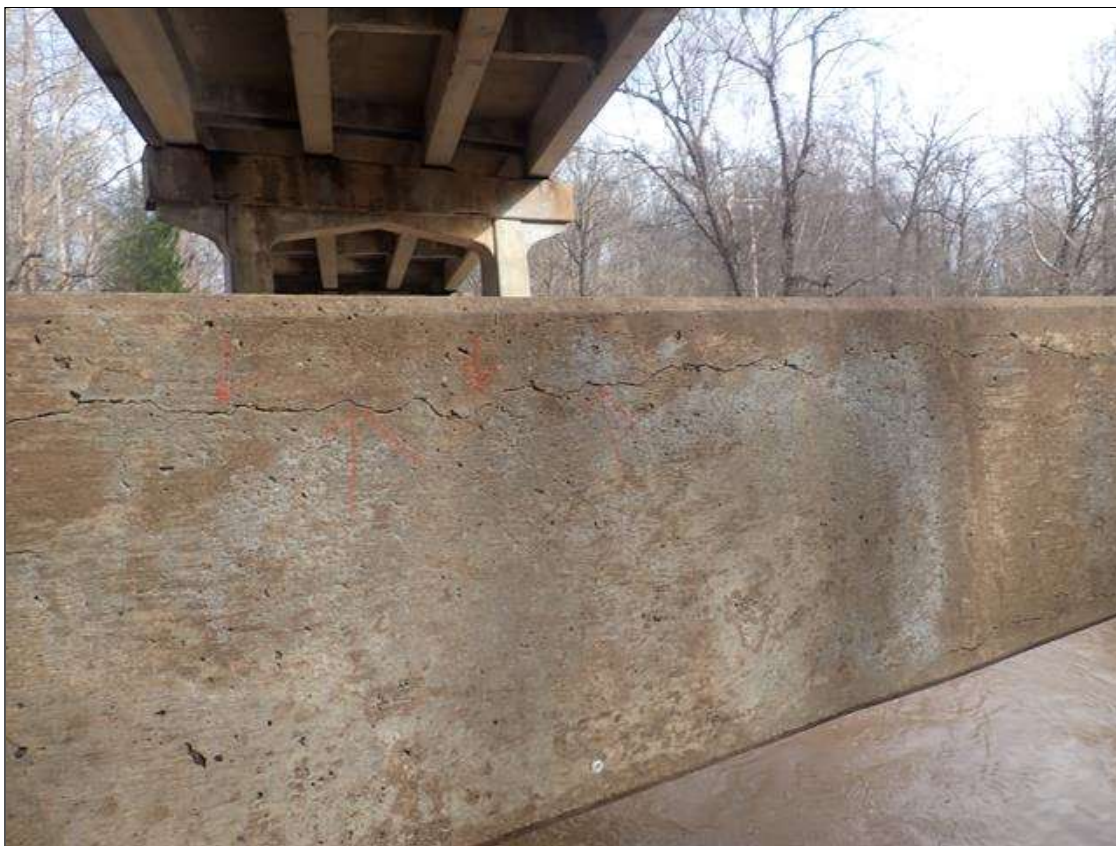
Bent 2 Pile 2: strut west face, horizontal crack (full length x up to 1/16in)
