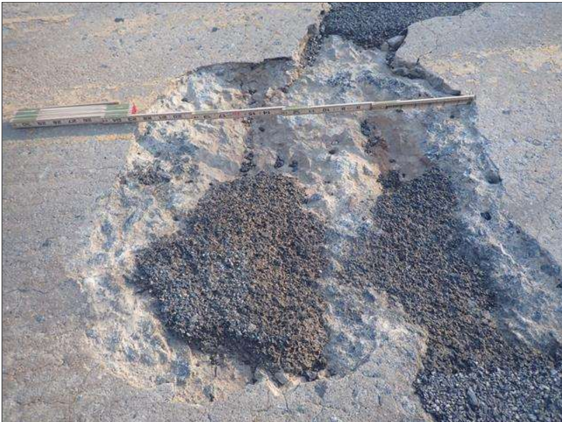
Span 3 Deck: (PAR) WESTBOUND LANE AT 9FT FROM BENT 2 JOINT, SPALL (30IN X 2FT X 2-1/2IN) WITH EXPOSED RUSTED REBARS
