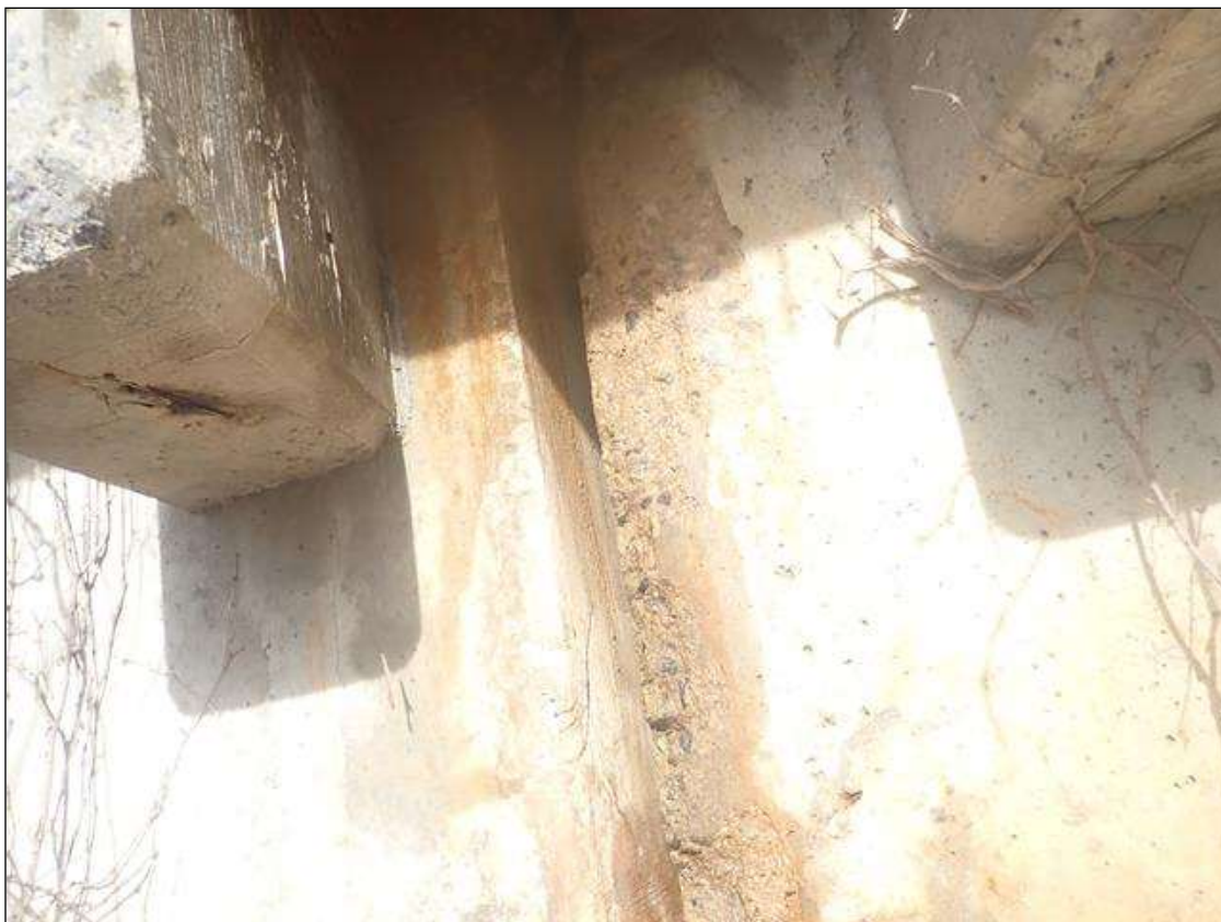
Span 5 Beam 4: 6 INCHES X 36 INCHES X UP TO 1-1/2 INCHES DEEP SPALL ON RIGHT SIDE OF WEB AT BENT 4 (PHOTO 1 OF 2)
