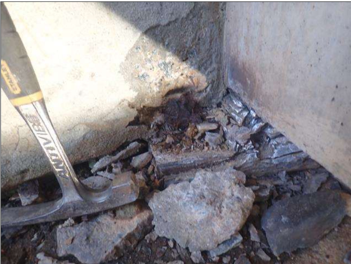
End Bent 2 Abutment: 22 INCHES X 12 INCHES AREA OF PATCH WITH 6 INCHES X 5 INCHES X 1 INCHES DEEP SPALL WITH EXPOSED REBAR AT NORTH END ADJACENT TO BEAM 1
