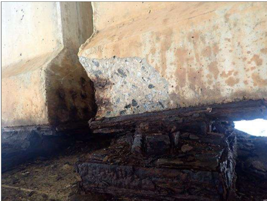
Span 2 Beam 2: (PAR) 9 INCHES X 7 INCHES X 2 1/2 INCHES DEEP SPALL WITH EXPOSED PRESTRESSING STRANDS ON LEFT SIDE OF BOTTOM FLANGE AT BENT 2
