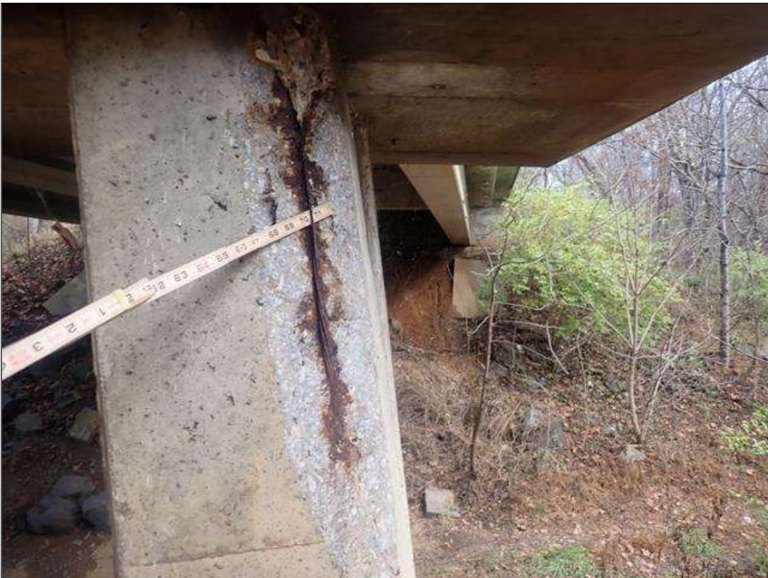
Bent 4 Row 1 Pile 5: (PAR) 31 INCHES X 5 INCHES X 5 INCHES DEEP SPALL WITH EXPOSED STRAND (UP TO 90% LOSS ON STRAND) ON SOUTHWEST CORNER
