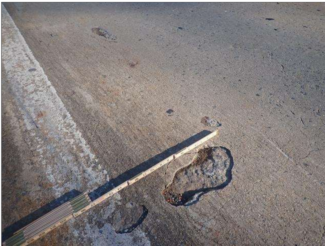
Span 1 Deck: both lanes scattered throughout, spalls (up to 10in x 6in x 1in) mainly at edges of previously patched area (photo 2 of 2)
