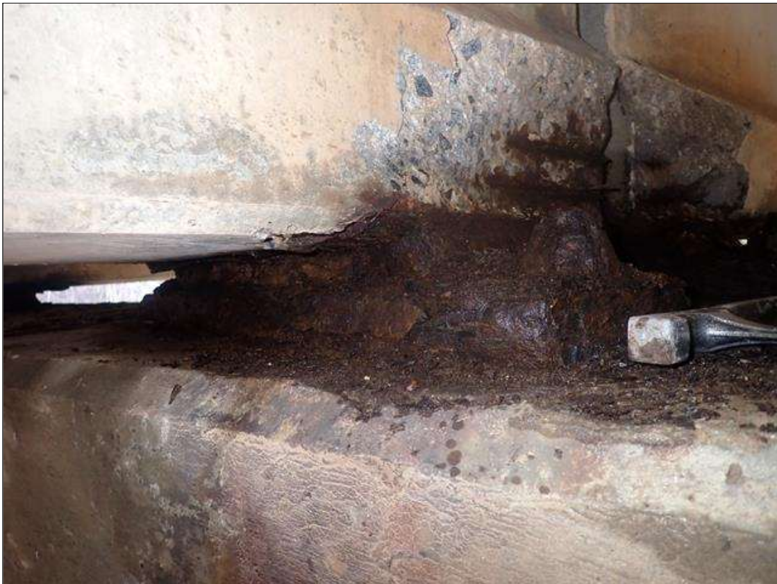
Span 3 Beam 2 - Far Bearing: RUST SCALE WITH SECTION LOSS (UP TO 1/8IN LOSS)
