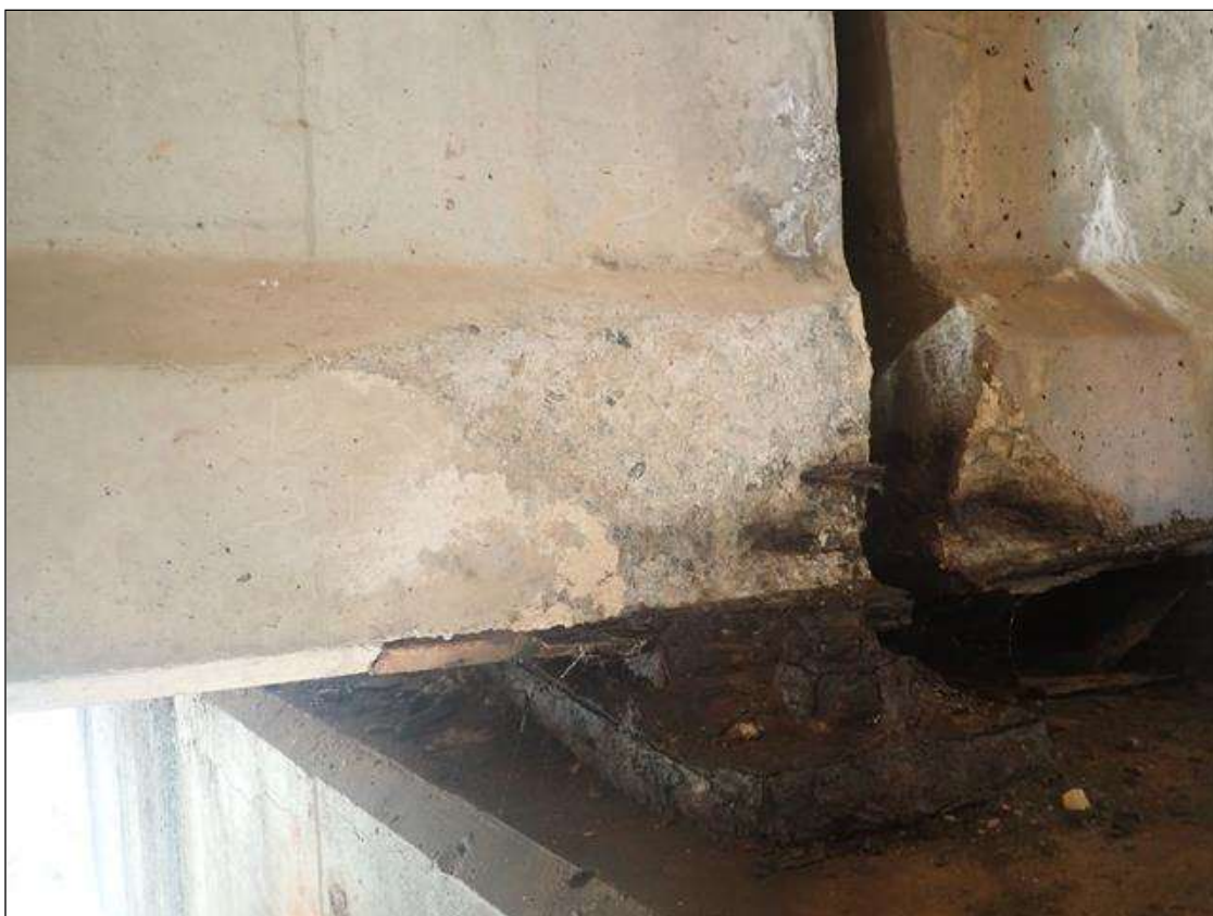
Span 5 Beam 3: (PAR) 16 INCHES X 9 INCHES X 2 INCHES DEEP SPALL WITH EXPOSED PRESTRESSING STRANDS ON LEFT SIDE OF BOTTOM FLANGE AT BENT 4
