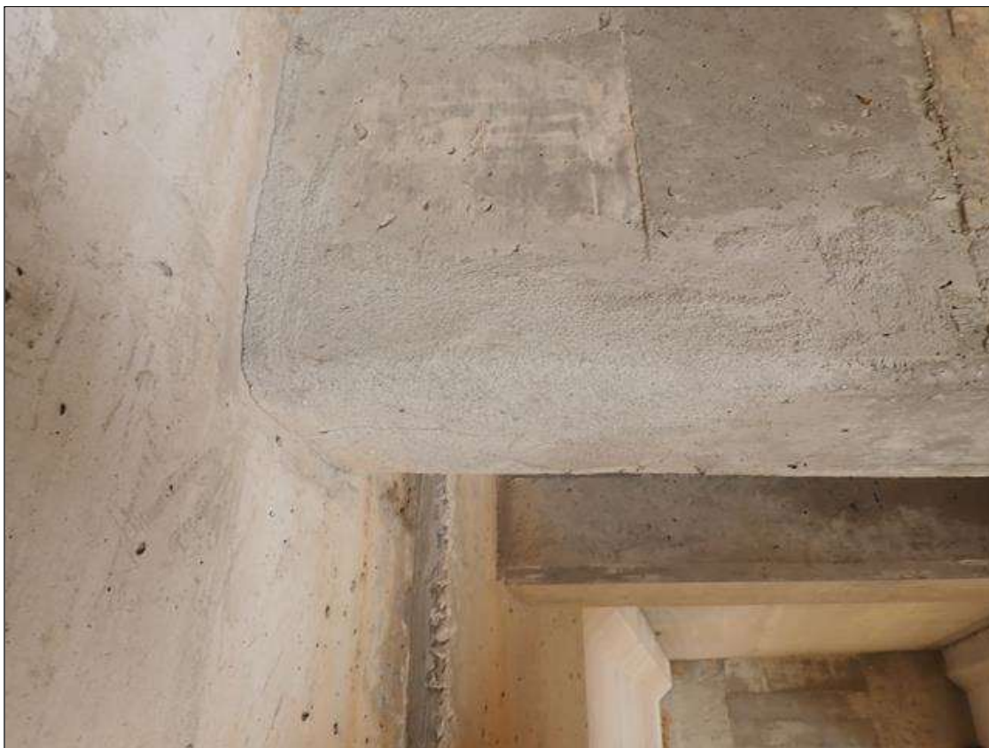
Span 3 Beam 1: 30 INCHES X 7 INCHES AREA OF SOUND PATCH ON BENT 3 DIAPHRAGM IN BAY 1
