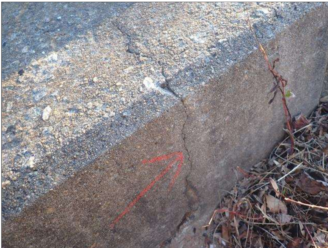
Span 1 Right Bridge Rail: (12 FEET X UP TO 1/32IN) LONGITUDINAL AND TRANSVERSE CRACKS ON CURB
