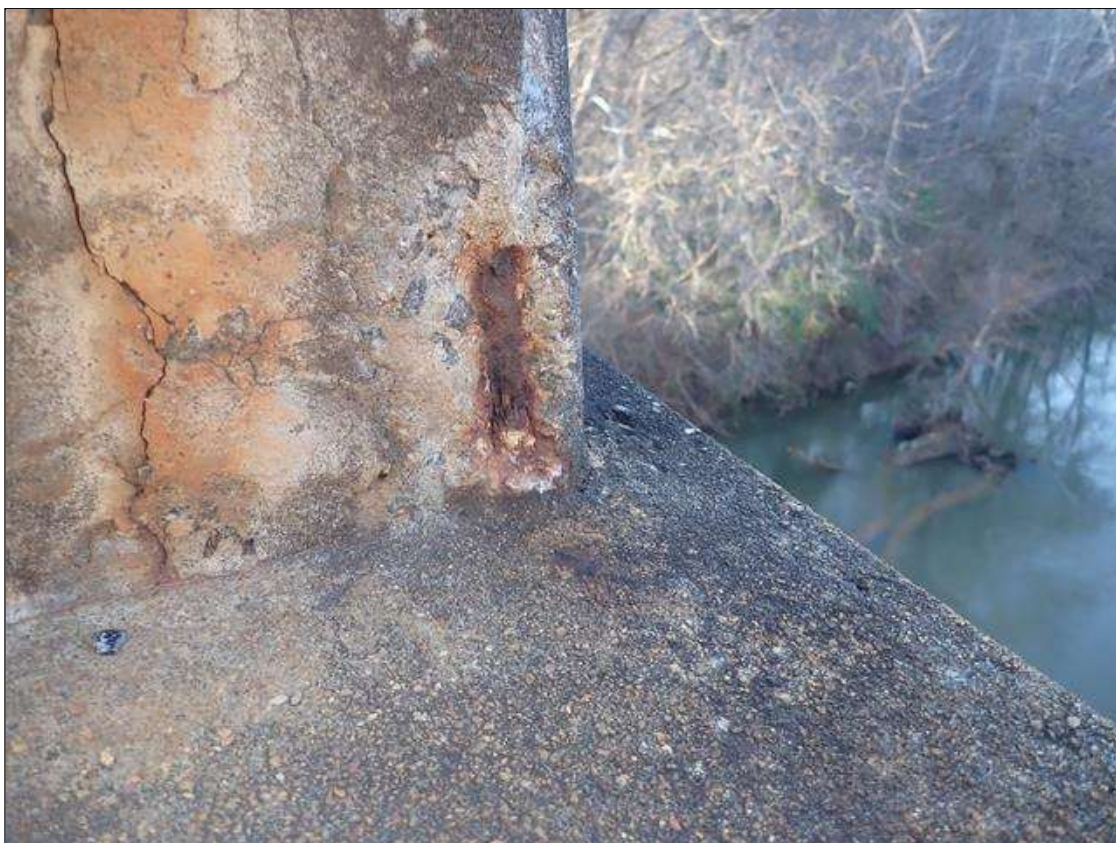
Span 3 Left Bridge Rail: 4 INCHES X 2 INCHES X 1/2 INCHES DEEP SPALL ON RAIL AT POST 1
