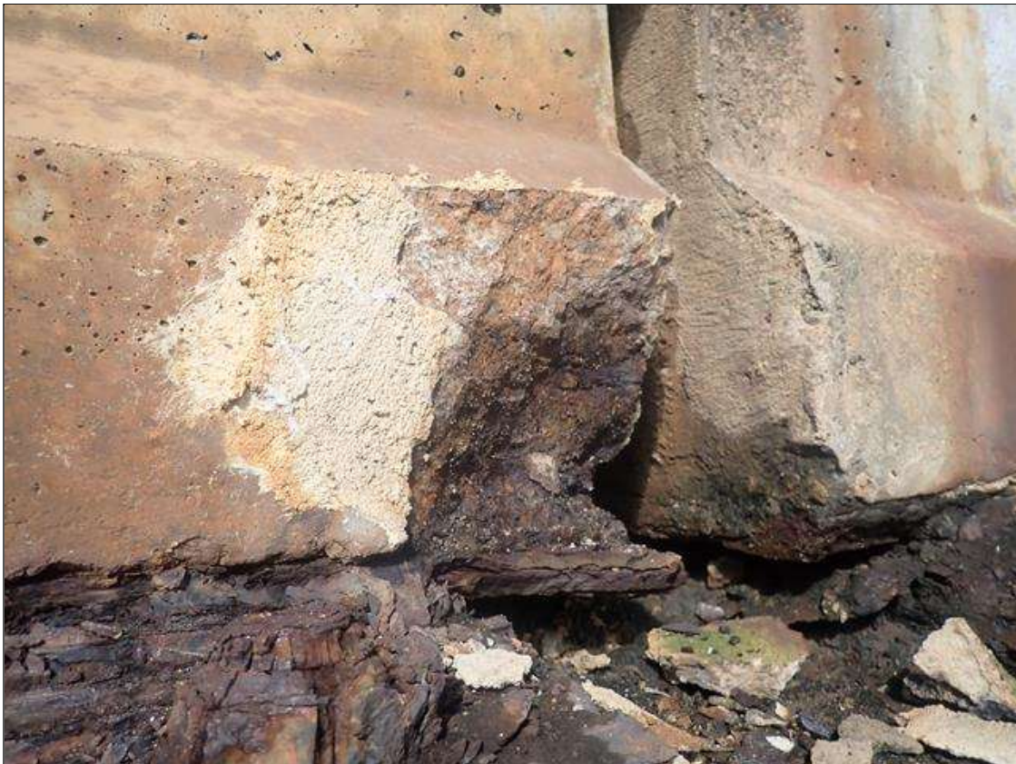
Span 3 Beam 4: (PAR) RIGHT SIDE OF BOTTOM FLANGE AT BENT 3, SPALL (17IN X 6IN X UP TO 2IN) WITH EXPOSED RUSTED STRANDS AT FAILED PATCHED AREA
