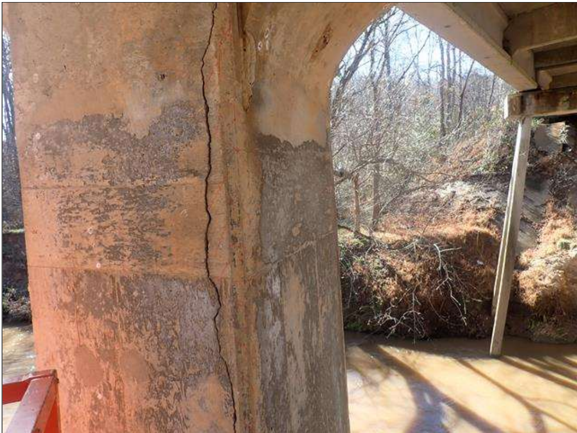
Bent 2 Pile 2: NORTHEAST CORNER AT 2FT BELOW CAP, DELAMINATION (5FT X 8IN)
