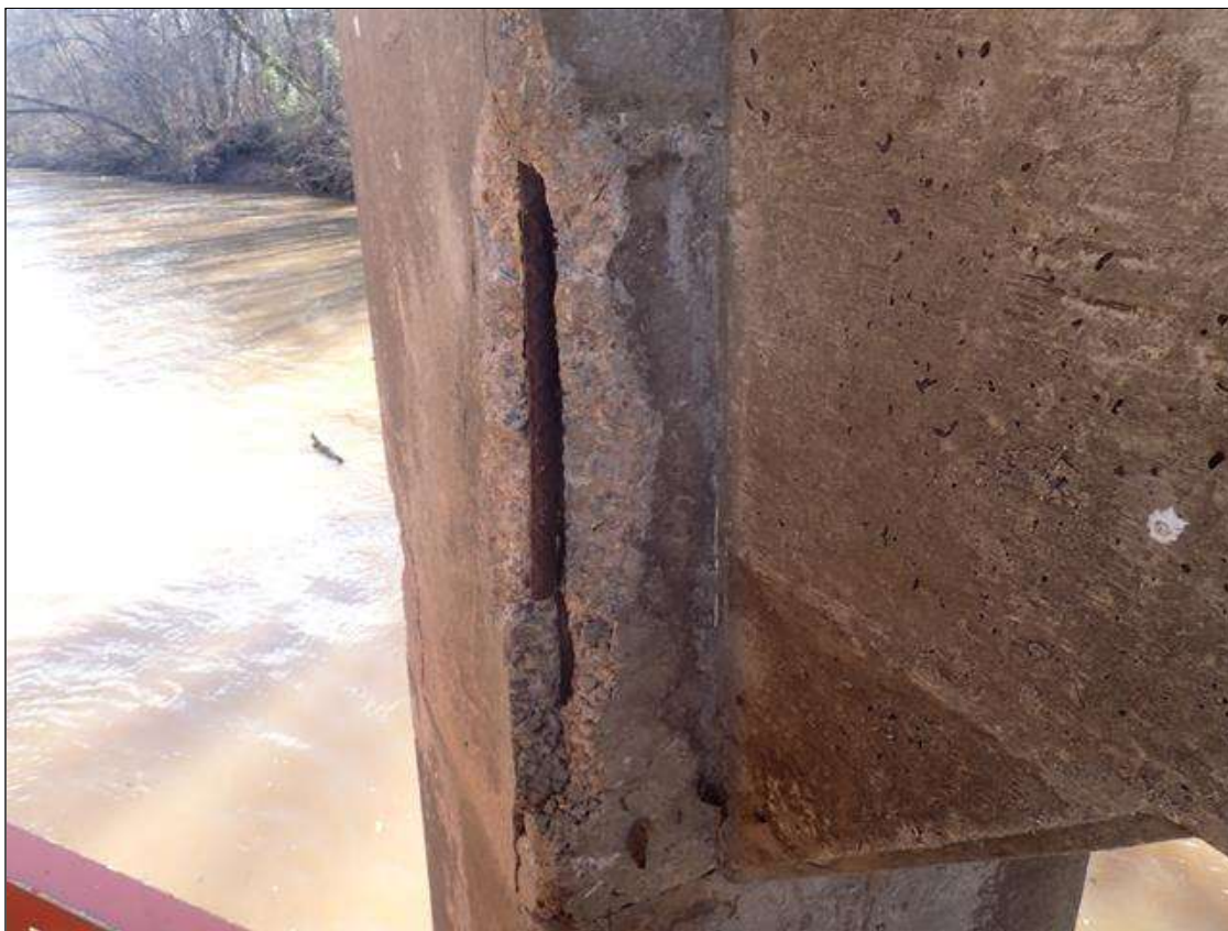
Bent 2 Pile 2: (PAR) 48 INCHES X 6 INCHES X 3-1/2 INCHES DEEP SPALL WITH EXPOSED REBAR ON NORTHEAST CORNER
