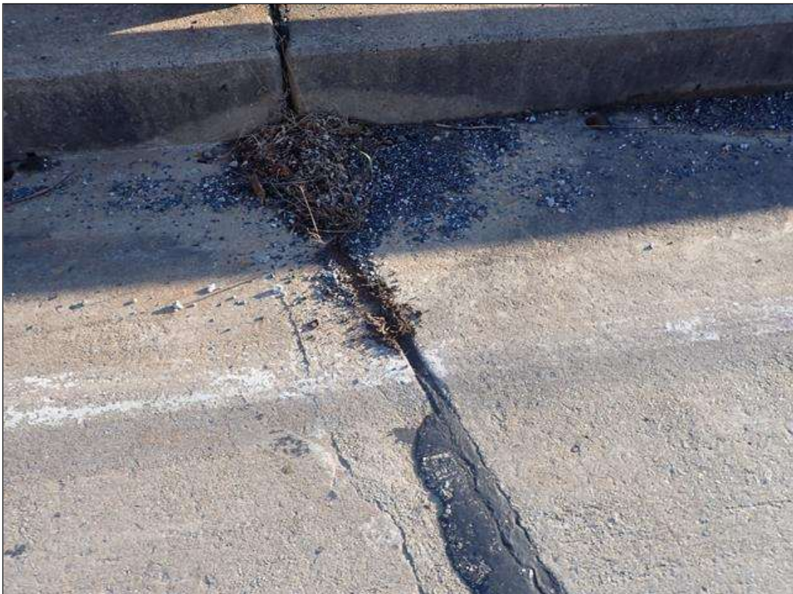
Span 5 Expansion Joint: 4 FEET DIRT AND DEBRIS IN SOUTH GUTTER
