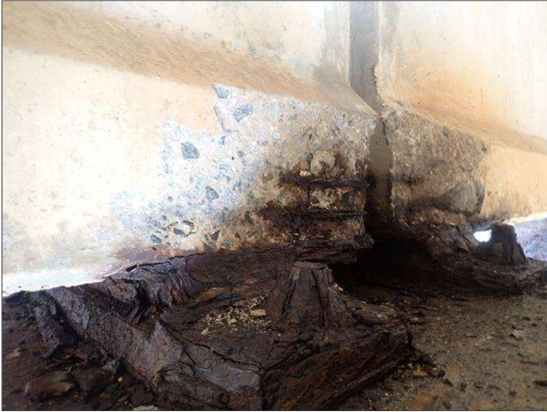
Span 3 Beam 2: (PAR) 16 INCHES X 8 INCHES X 2 INCHES DEEP SPALL WITH EXPOSED PRESTRESSING STRANDS ON RIGHT SIDE OF BOTTOM FLANGE AT BENT 3
