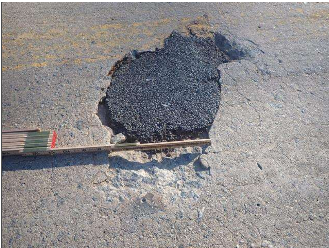
Span 1 Deck: both lanes scattered throughout, spalls (up to 10in x 6in x 1in) mainly at edges of previously patched area (photo 1 of 2)
