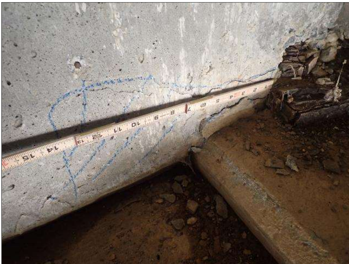
End Bent 1 Abutment: 14 INCHES X 8 INCHES AREA OF DELAMINATION IN BAY 3 ADJACENT TO BEAM 3
