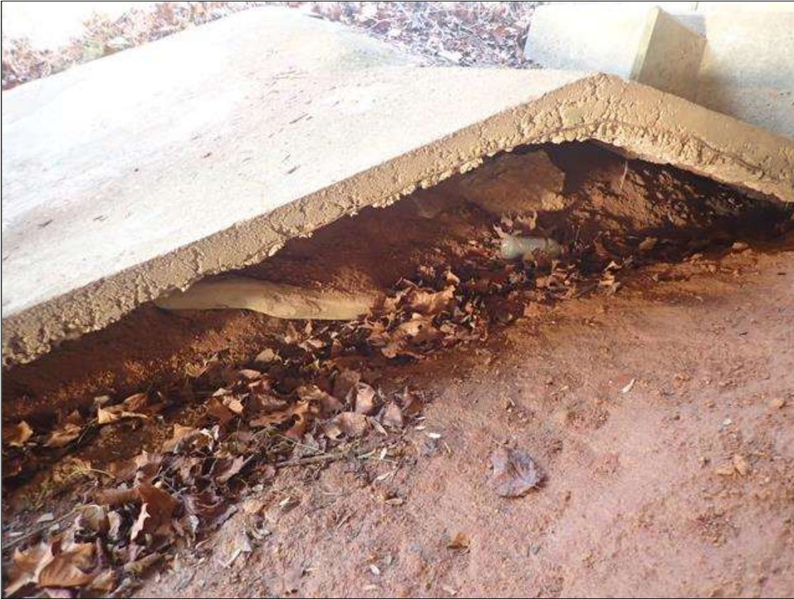
Slope Protection: end bent 2 slope protection north end, erosion with undermining (12ft x 2ft x full width)
