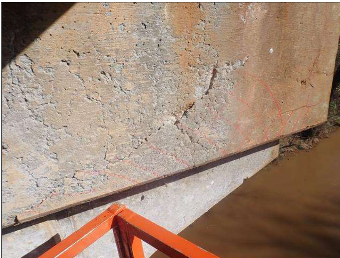
Bent 3 Cap 1: 5FT X 15 INCHES AREA OF DELAMINATION ON WEST FACE UNDER BEAM 4
