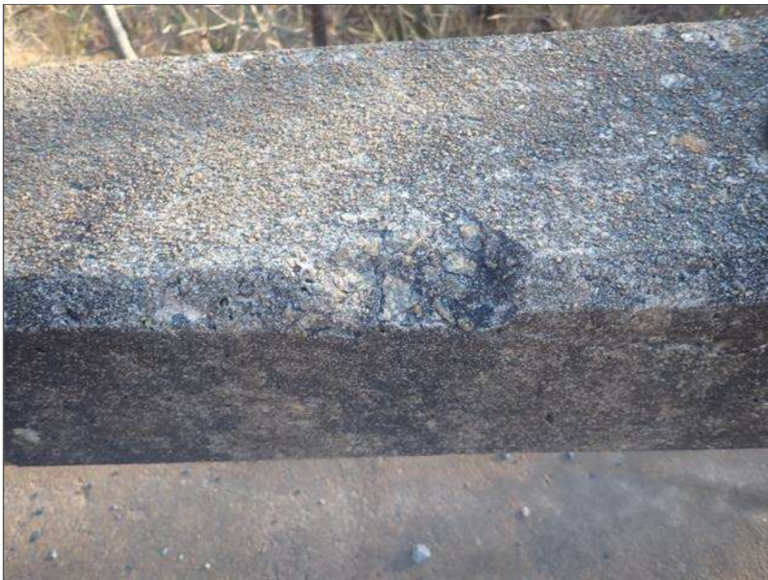
Span 5 Right Bridge Rail: 4 INCHES X 3 INCHES X 1/2 INCHES DEEP SPALL ON RAIL NEAR POST 5
