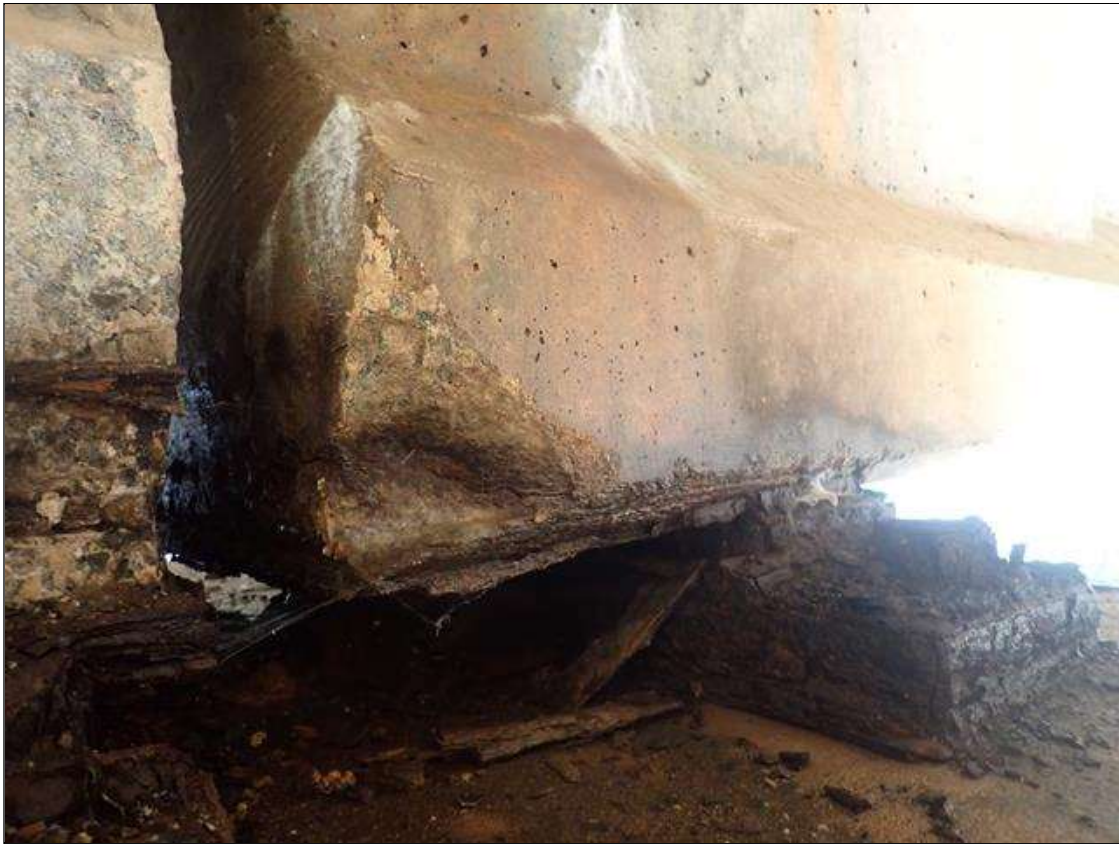
Span 4 Beam 3: LEFT SIDE OF BOTTOM FLANGE SPLIT AT BENT 4, SPALL (6IN X 6IN X 1-1/2IN) WITH RUST STAINING
