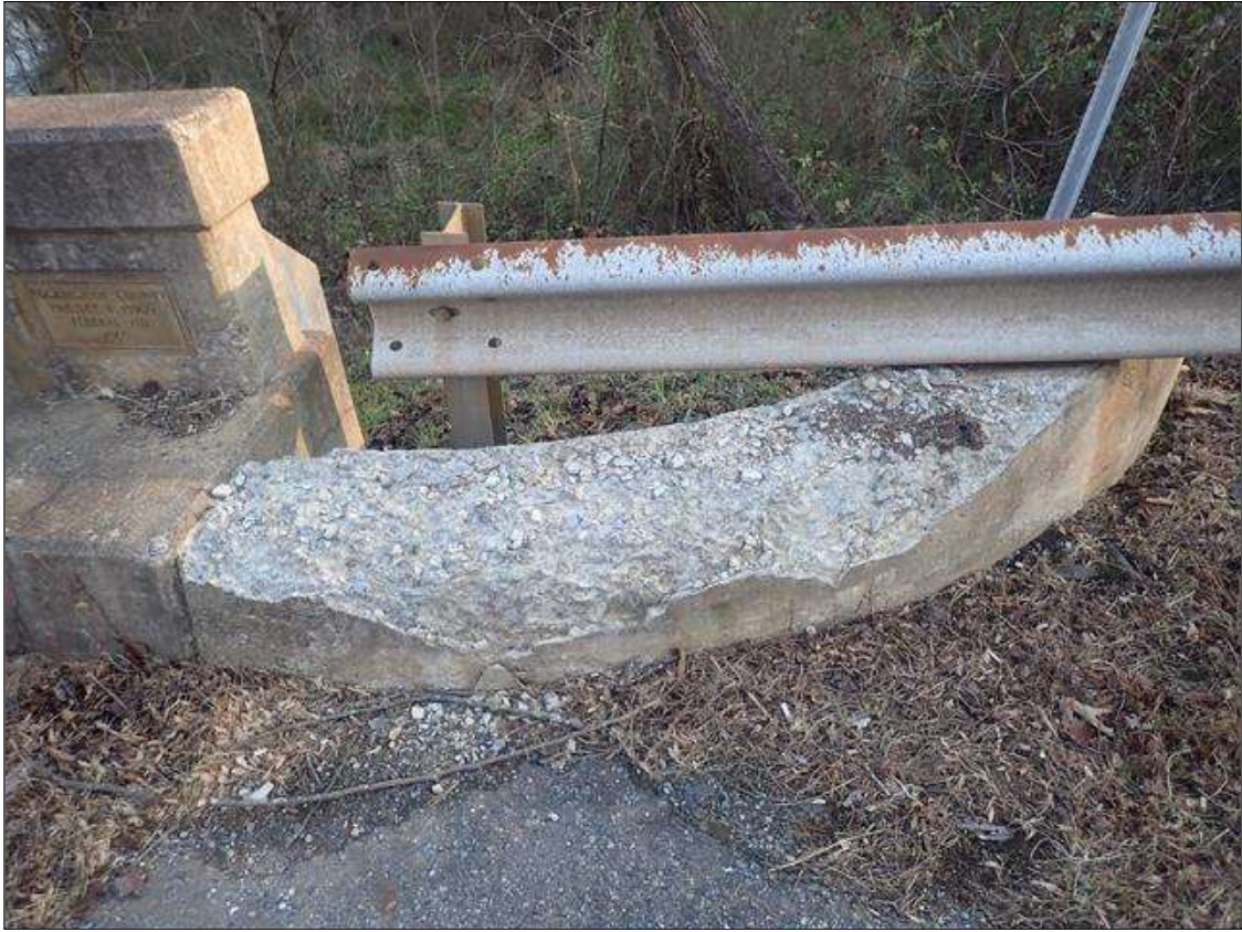
Span 1 Right Bridge Rail: RAIL EXTENSION AT END BENT 1, SPALL (6-1/2FT X FULL WIDTH X UP TO 1IN)
