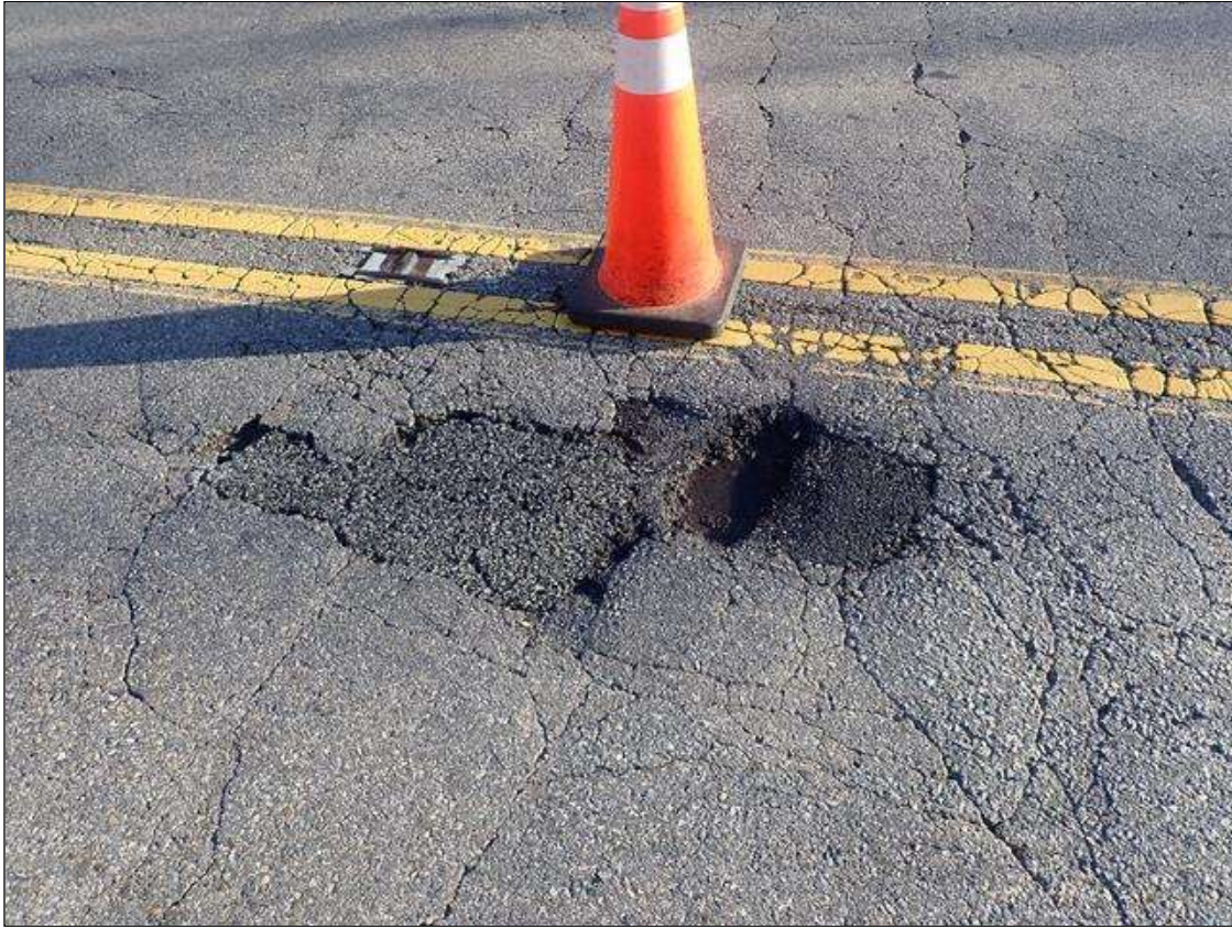
General Comments and Misc Items: west approach westbound lane at 9ft from end bent 1, pothole (9in x 15in x 3in)
