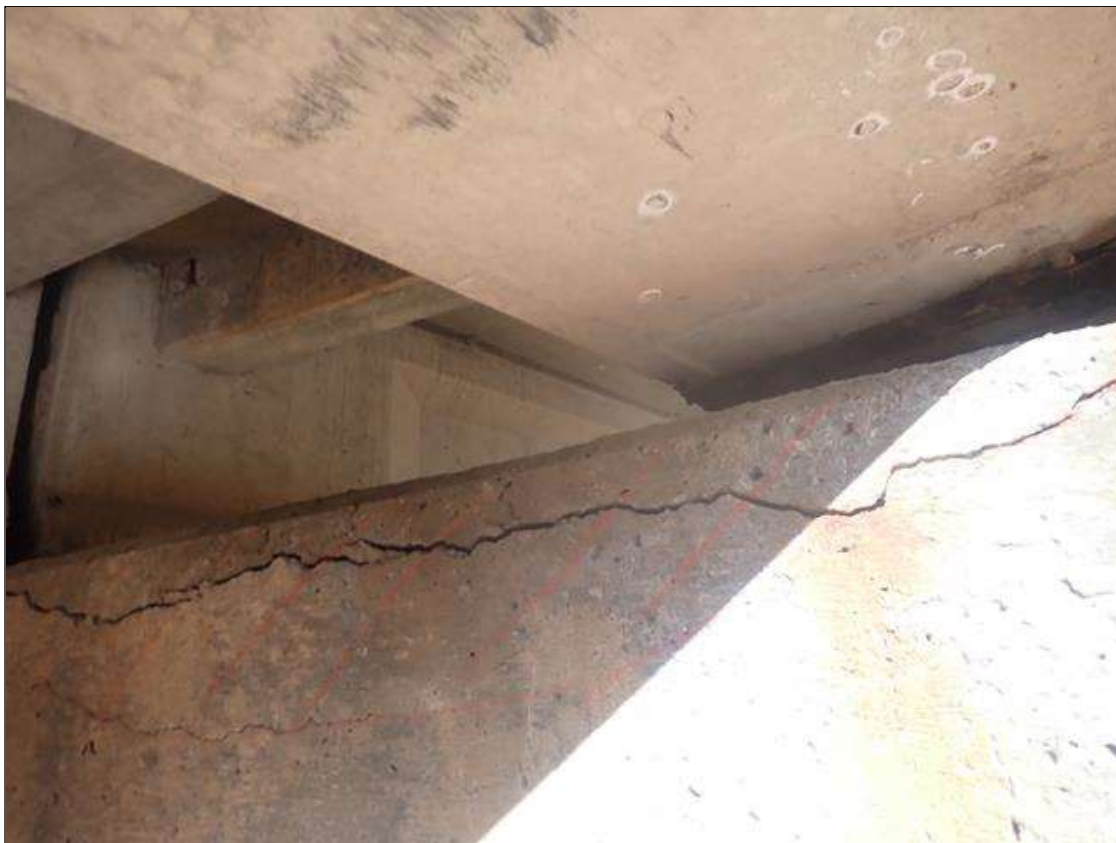
Bent 3 Cap 1: 6-1/2FT X UP TO 9IN DELAMINATION ON WEST FACE UNDER BAY 3
