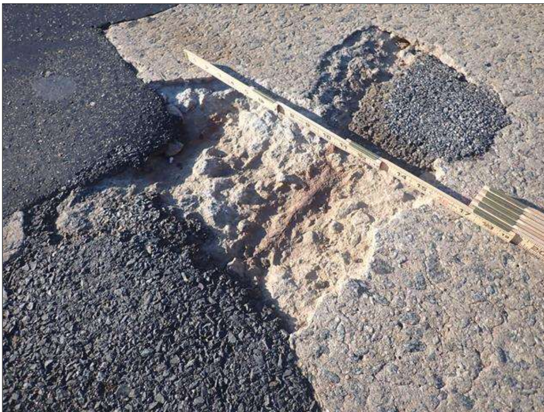
Span 4 Deck: (PAR) EASTBOUND LANE AT 9FT FROM BENT 3 JOINT, SPALL (2FT X 16IN X UP TO 2IN) WITH EXPOSED RUSTED REBARS
