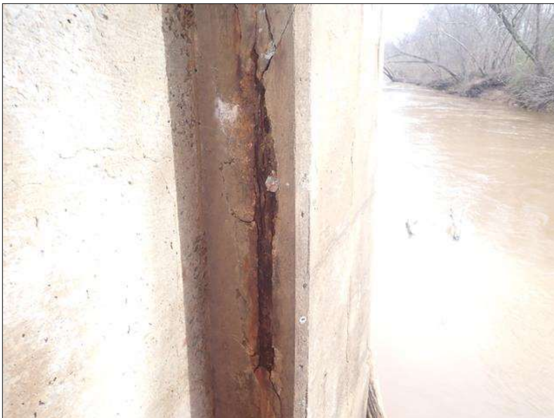
Bent 2 Pile 2: (PAR) 32 INCHES X 4 INCHES X 1 INCHES DEEP SPALL WITH EXPOSED REBAR ON NORTH FACE
