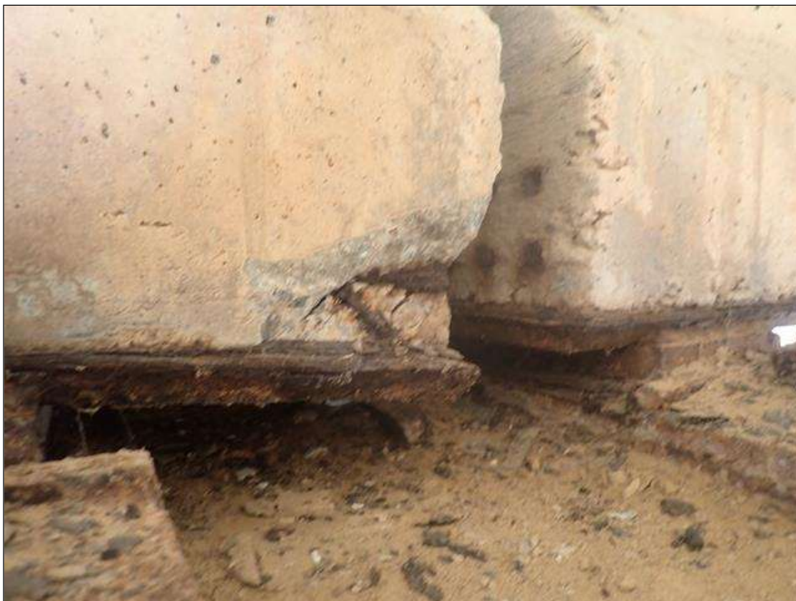
Span 3 Beam 3: (PAR) 5 1/2 INCHES X 3 INCHES X 2 INCHES DEEP SPALL WITH EXPOSED PRESTRESSING STRANDS ON RIGHT SIDE OF BOTTOM FLANGE AT BENT 3
