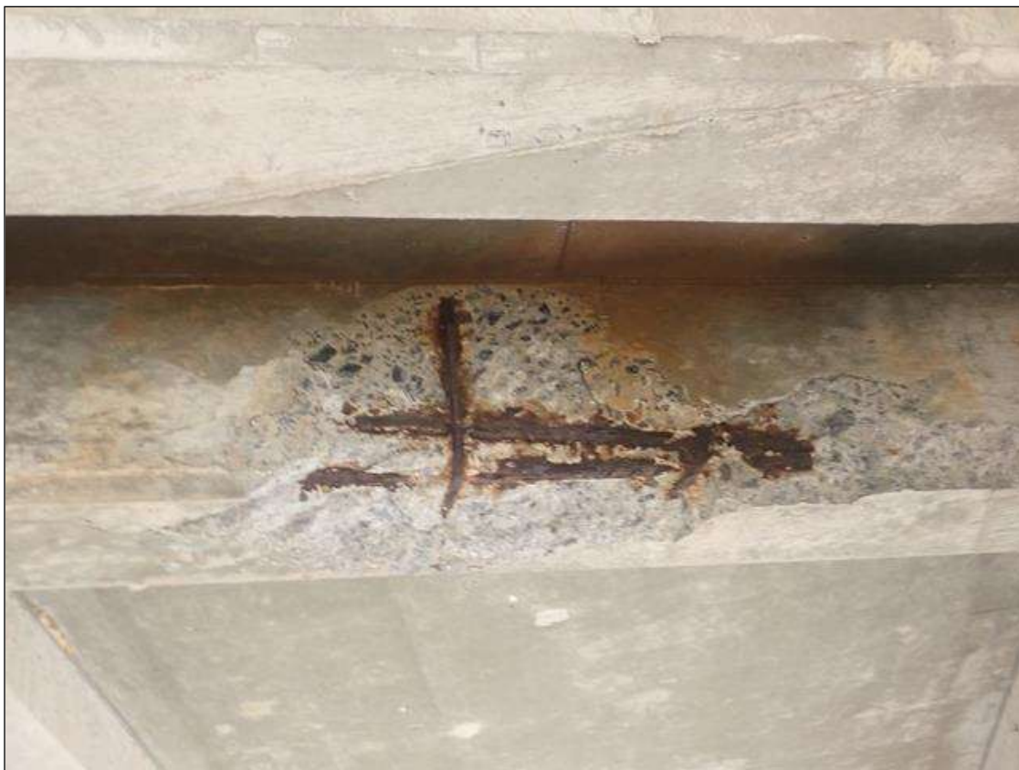
Span 5 Beam 2: 40 INCHES X 18 INCHES X 3 INCHES DEEP SPALL WITH EXPOSED REBAR ON BENT 4 DIAPHRAGM IN BAY 1
