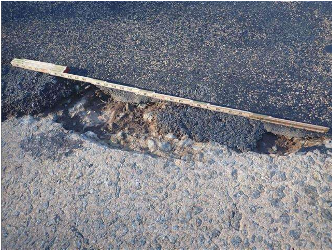
Span 2 Deck: (PAR) 30 INCHES X 12 INCHES X 2 INCHES DEEP SPALL WITH EXPOSED REBAR AND AREA OF DELAMINATION IN EASTBOUND LANE, 11 FEET FROM BENT 1
