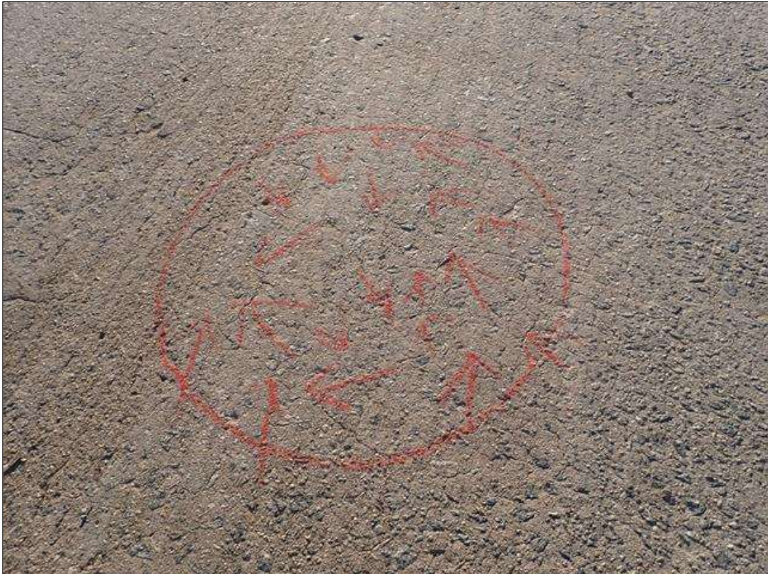
Span 5 Deck: 900 SQUARE FEET HAIRLINE MAP CRACKING
