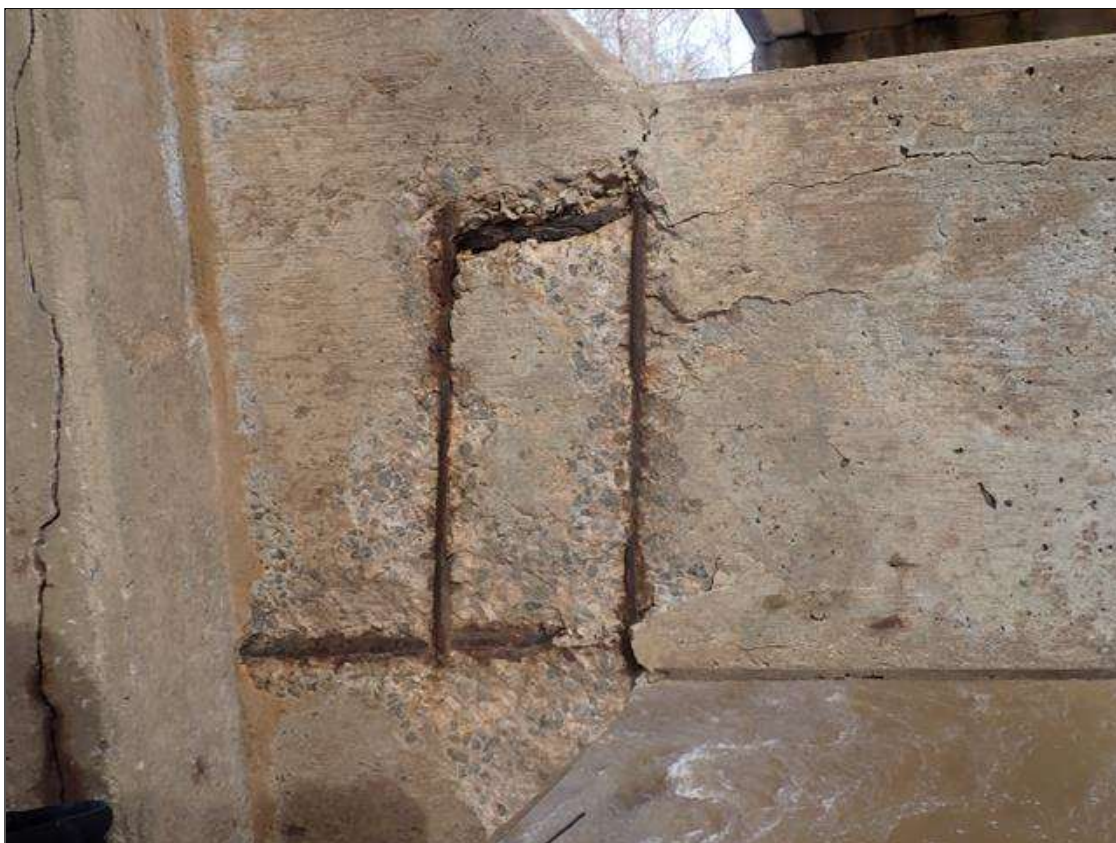
Bent 2 Pile 1: 32 INCHES X 30 INCHES X 1 1/2 INCHES DEEP SPALL WITH EXPOSED REBAR ON WEST FACE OF STRUT
