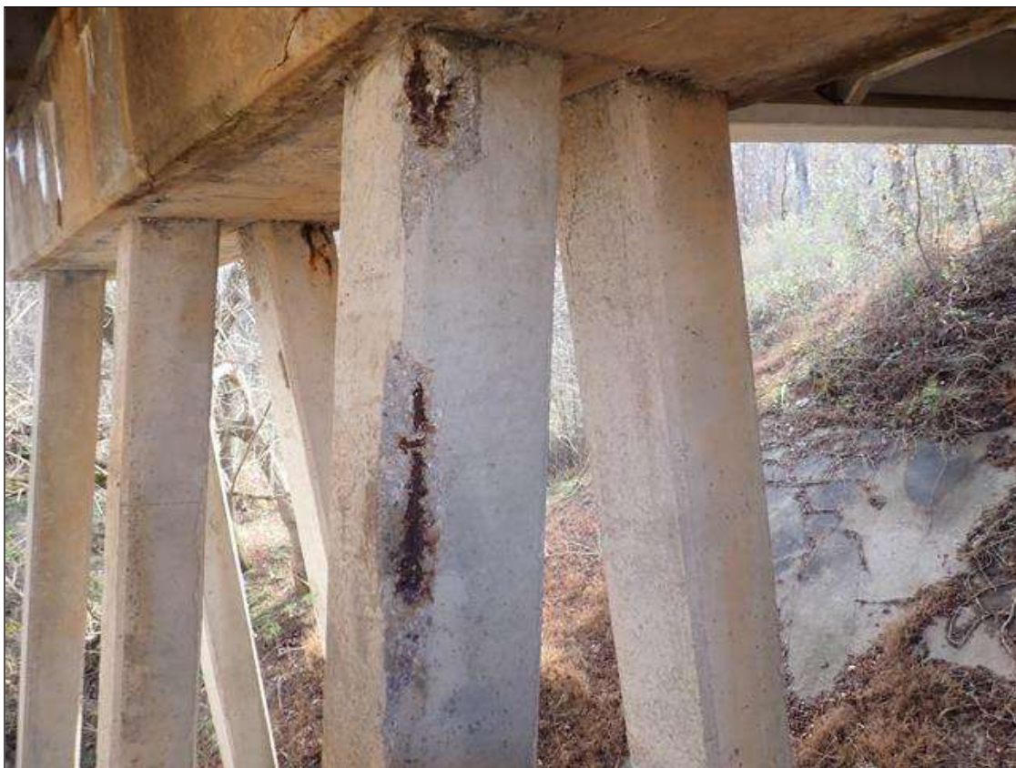
Bent 1 Row 2 Pile 3: (PAR) EAST FACE BELOW CAP, (2) SPALL/DELAMINATION (UP TO 27IN X 5IN X 2IN) WITH EXPOSED RUSTED STRAND
