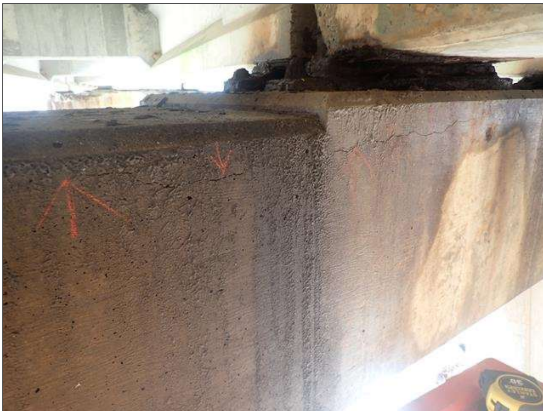
Bent 4 Cap 1: EAST FACE BELOW BEAM 3, HORIZONTAL CRACK (35IN X UP TO 1/16IN)
