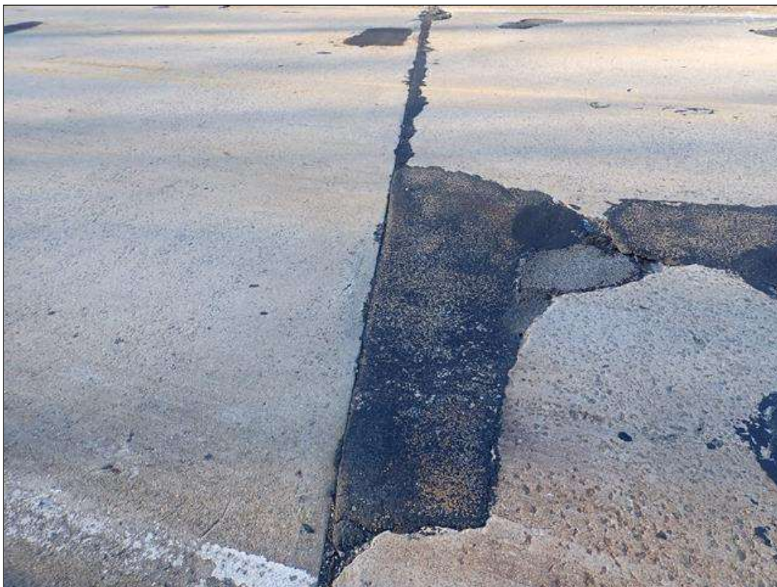
Span 2 Expansion Joint: (NOT OBSERVED AS OF 2022-11-18) 10 INCHES X 6 INCHES X 2 1/2 INCHES DEEP SPALL WITH EXPOSED REBAR IN EASTBOUND LANE ALONG BENT 1 JOINT
