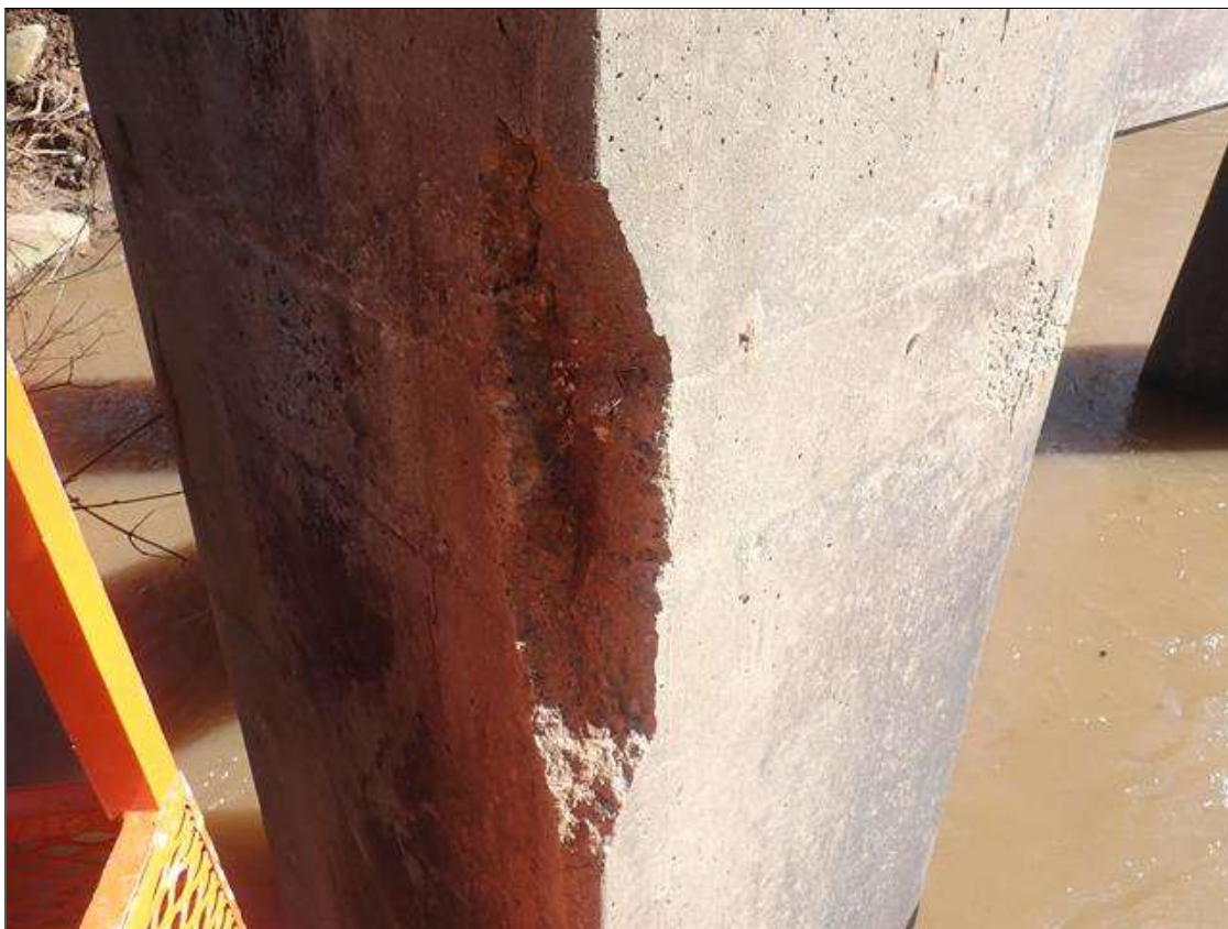
Bent 3 Pile 1: (PAR) 36 INCHES X 6 INCHES X 2 INCHES DEEP SPALL WITH EXPOSED REBAR AT NORTHWEST CORNER
