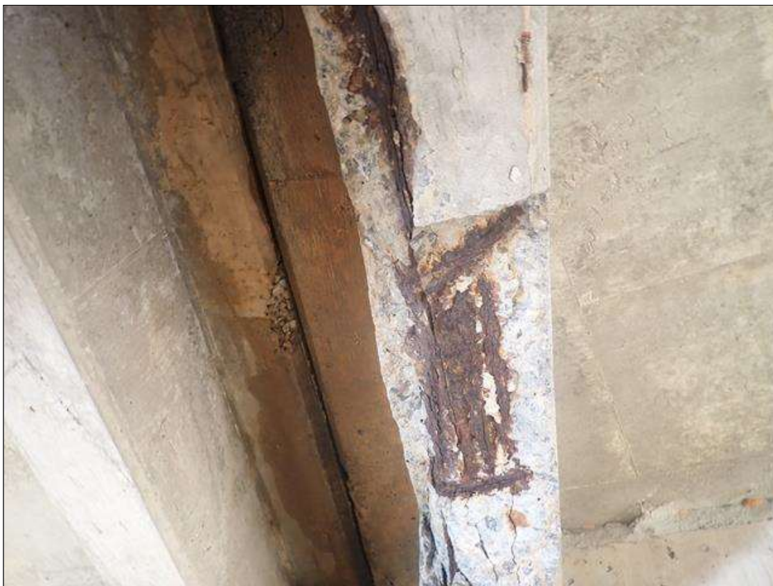
Span 3 Beam 3: 89 INCHES X 10 INCHES X 7 INCHES DEEP SPALL WITH EXPOSED REBAR ON BENT 2 DIAPHRAGM IN BAY 2
