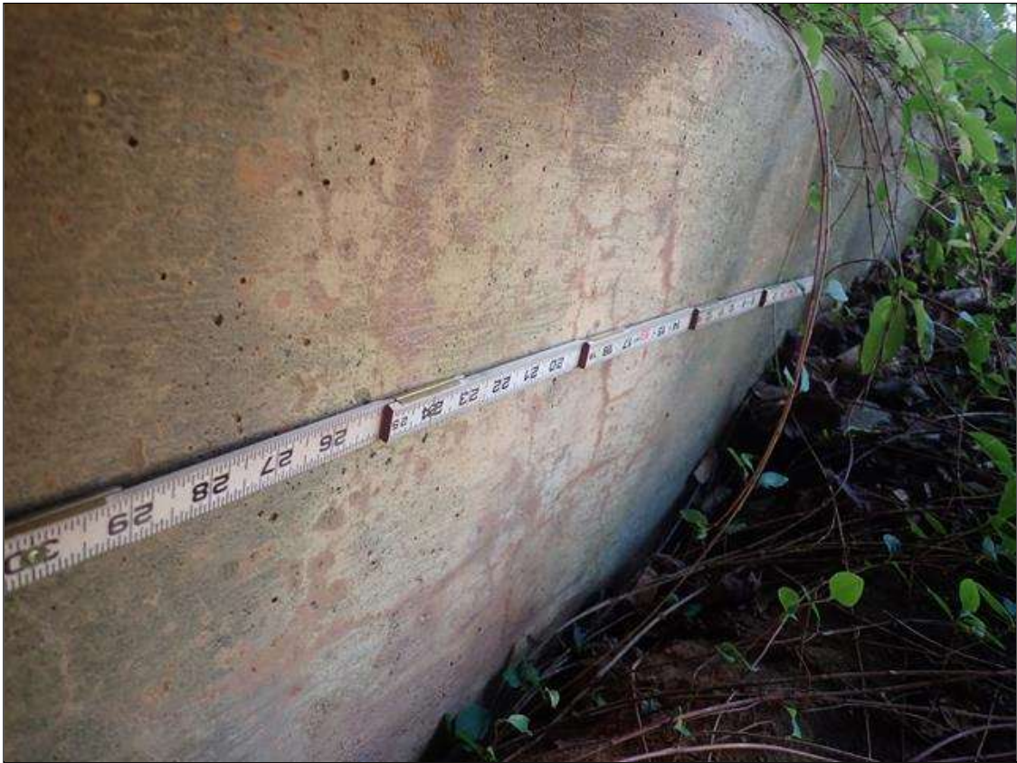
End Bent 1 Cap 1: 30 INCHES X 12 INCHES AREA OF HAIRLINE MAP CRACKING UNDER BEAM 1
