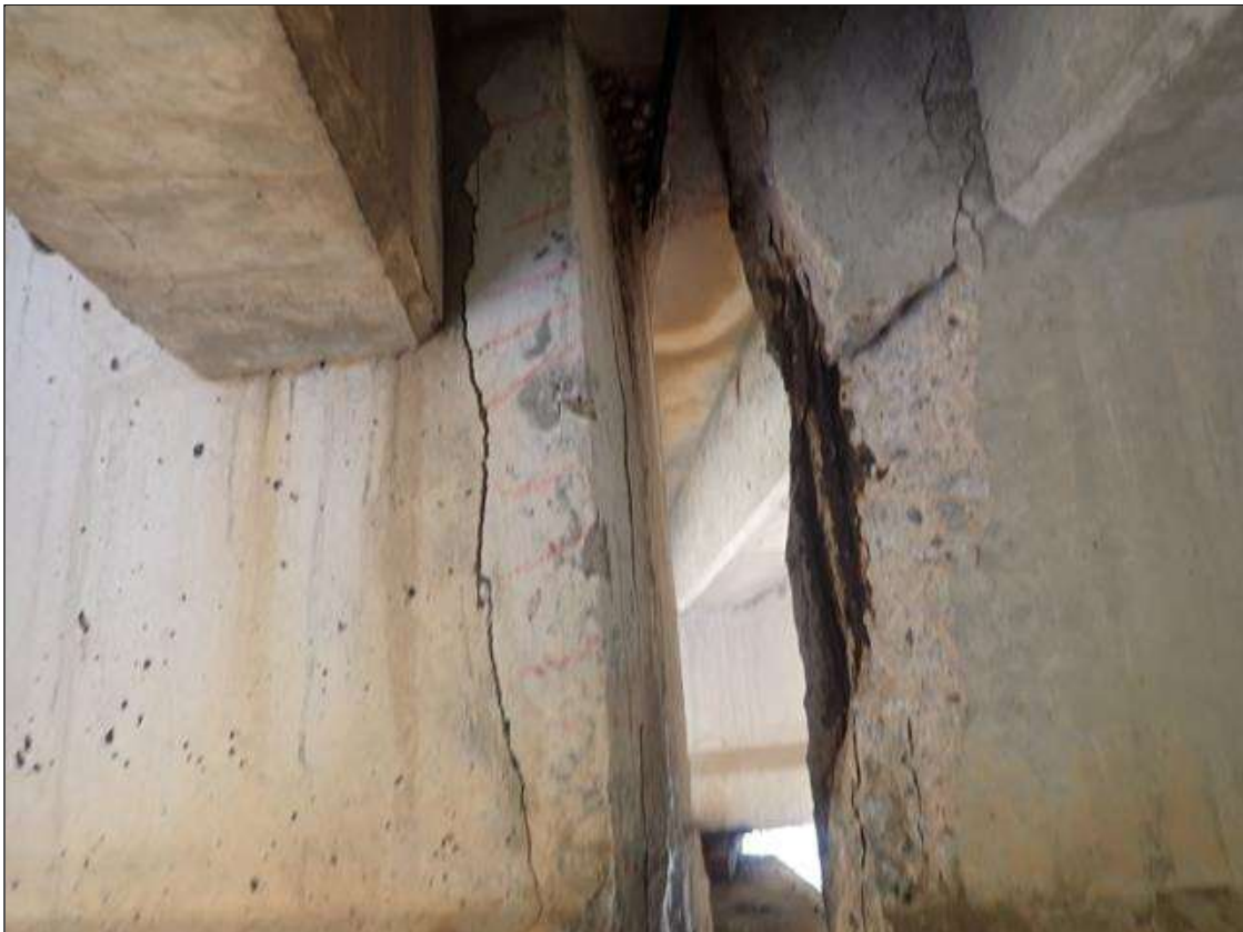
Span 2 Beam 3: 7 INCHES X 36 INCHES AREA OF DELAMINATION WITH 1/8 INCHES VERTICAL CRACK ON LEFT SIDE OF WEB AT BENT 1
