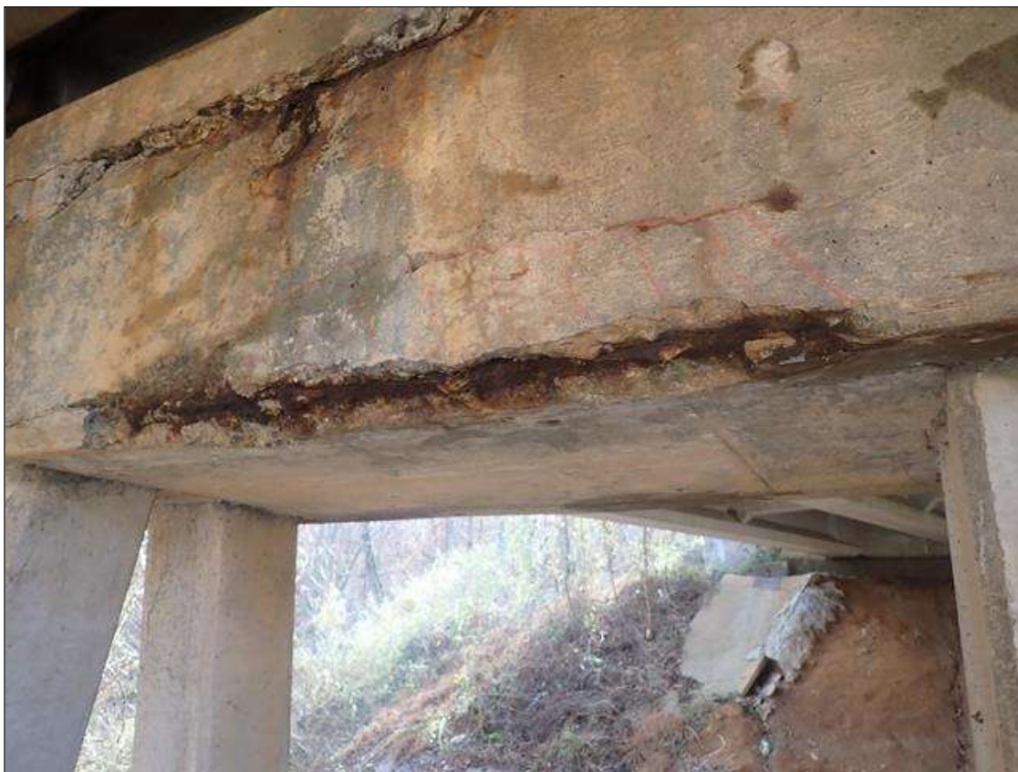
Bent 1 Cap 1: (PAR) EAST FACE BETWEEN PILES 2 AND 3, SPALL/DELMINATION (6FT X UP TO 10IN X 2-1/2IN) WITH EXPOSED RUSTED REBAR
