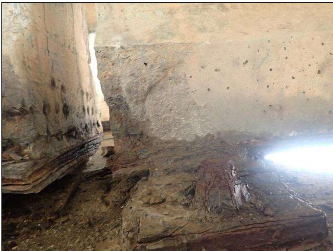
Span 3 Beam 3: (PAR) 7 INCHES X 7 INCHES X 2 1/2 INCHES DEEP SPALL WITH EXPOSED PRESTRESSING STRANDS ON RIGHT SIDE OF BOTTOM FLANGE AT BENT 2
