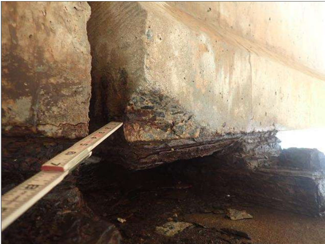
Span 4 Beam 2: (PAR) BOTTOM FLANGE LEFT SIDE AT BENT 4, SPALL (8IN X 4IN X 2IN) WITH EXPOSED PRESTRESSING STRAND
