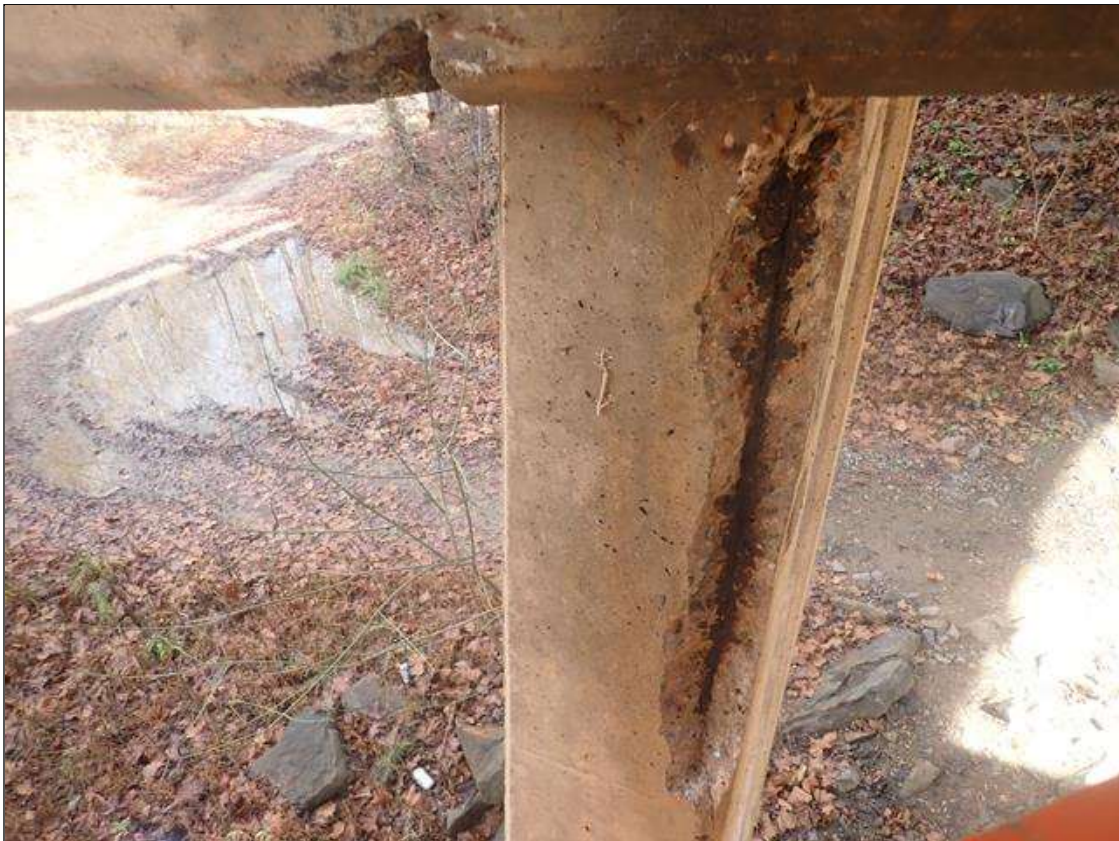
Bent 4 Row 1 Pile 1: (PAR) SOUTHWEST CORNER BELOW CAP, SPALL (3FT X 4IN X 2IN) WITH EXPOSED RUSTED STRAND
