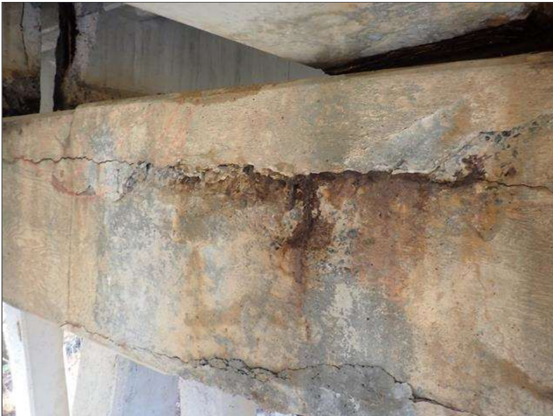
Bent 1 Cap 1: (PAR) 60 INCHES X 5 INCHES X 3 INCHES DEEP AND 48 INCHES X 10 INCHES X 2 INCHES DEEP SPALL WITH EXPOSED REBAR ON EAST FACE UNDER BEAM 2
