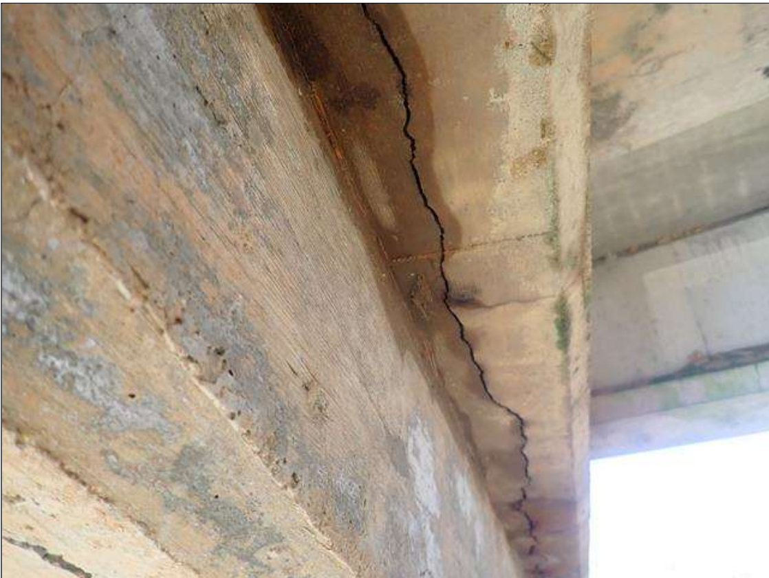
Bent 3 Cap 1: (19 FEET X UP TO 1/8 INCHES) TRANSVERSE CRACK WITH RUST STAINING ON BOTTOM OF CAP
