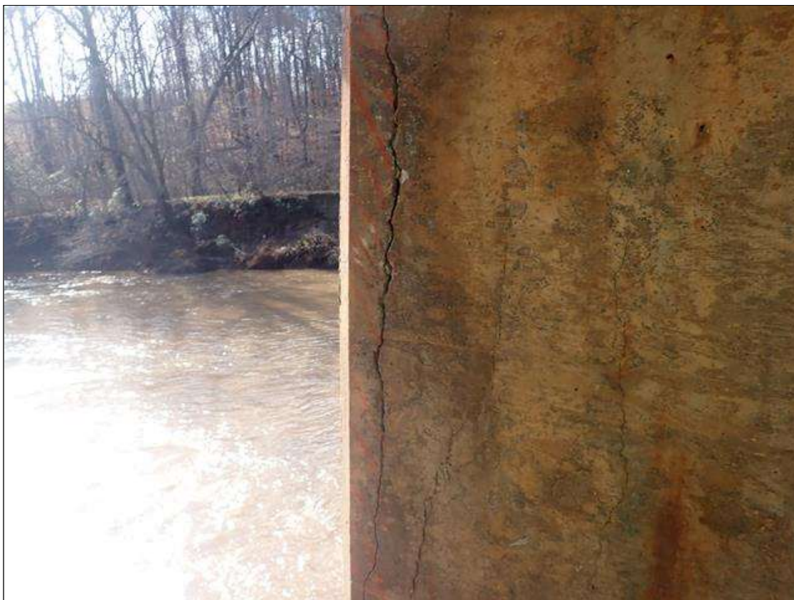
Bent 3 Pile 2: 7 FEET X 8 INCHES AREA OF DELAMINATION WITH 1/8 INCHES VERTICAL CRACK ON SOUTHEAST CORNER
