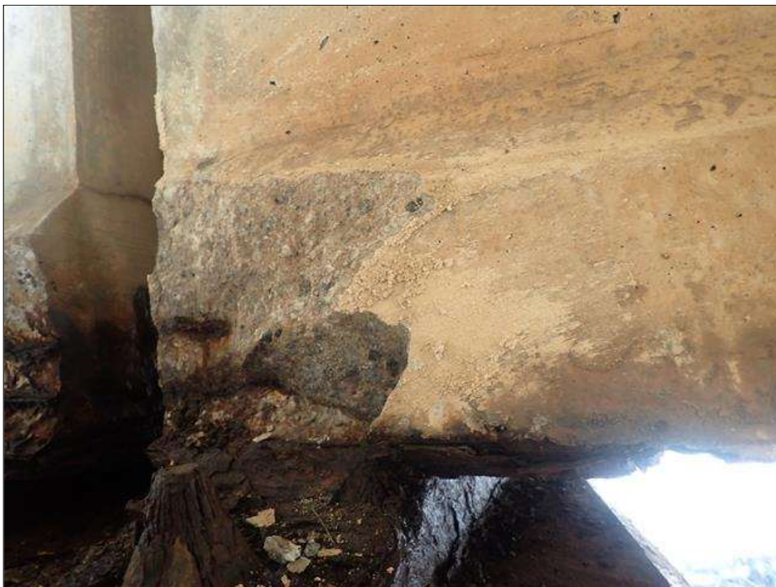
Span 4 Beam 2: (PAR) 11 INCHES X 9 INCHES X 2 INCHES DEEP SPALL WITH EXPOSED PRESTRESSING STRANDS ON RIGHT SIDE OF BOTTOM FLANGE AT BENT 3
