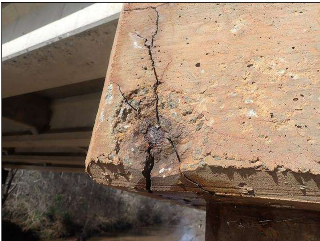
Bent 3 Cap 1: 6 INCHES DIAMETER X 1 INCHES DEEP SPALL WITH EXPOSED REBAR ON SOUTH FACE
