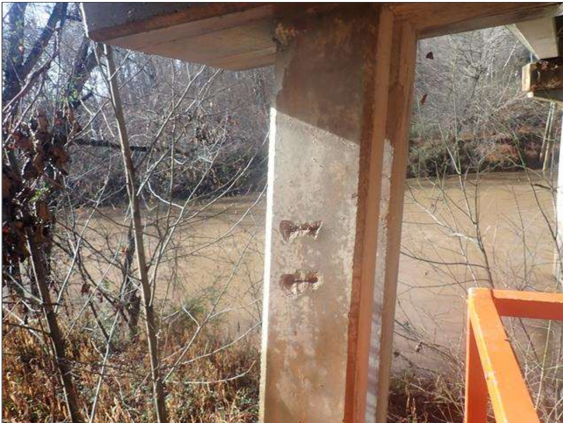
Bent 4 Row 2 Pile 5: EAST FACE BELOW CAP, (3) SPALLS (UP TO 9IN X 4IN X 1-1/2IN) WITH EXPOSED RUSTED REBAR
