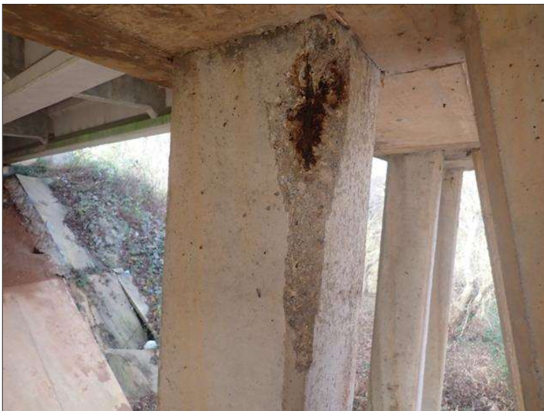
Bent 1 Row 1 Pile 3: (PAR) SOUTHEAST CORNER BELOW CAP, SPALL(21IN X 6IN X 2IN) WITH EXPOSED RUSTED STRAND
