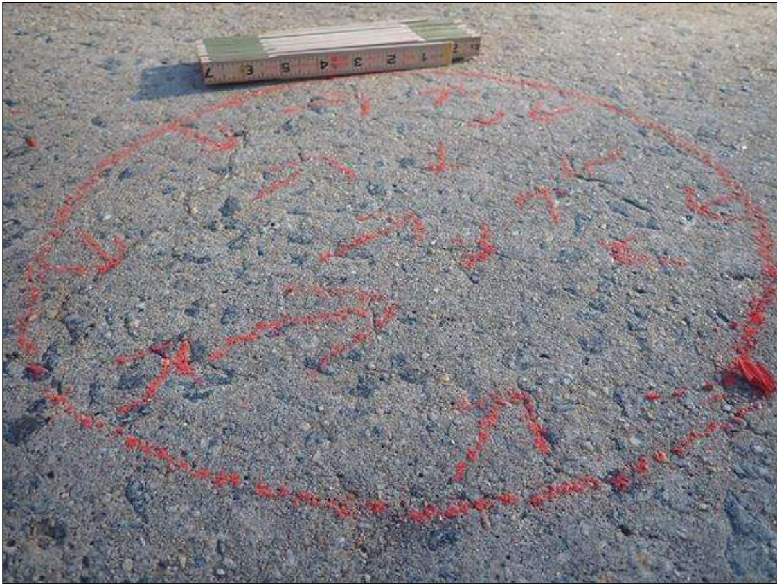
Span 1 Deck: 1008 SQUARE FEET HAIRLINE MAP CRACKING
