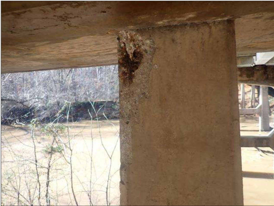
Bent 4 Row 2 Pile 3: (PAR) SOUTHEAST CORNER BELOW CAP, SPALL (16IN X 4-1/2IN X 2IN) WITH EXPOSED RUSTED STRAND
