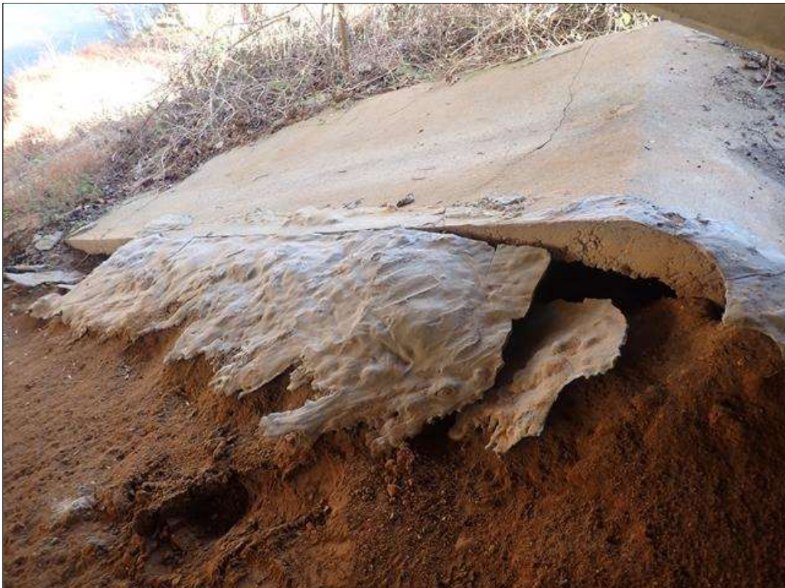
Slope Protection: end bent 1 slope protection under beam 4, failed repair with erosion causing undermining (up to 2ft x up to 1ft deep x full width) of the slope at top and below intermediate diaphragm (photo 2 of 2)
