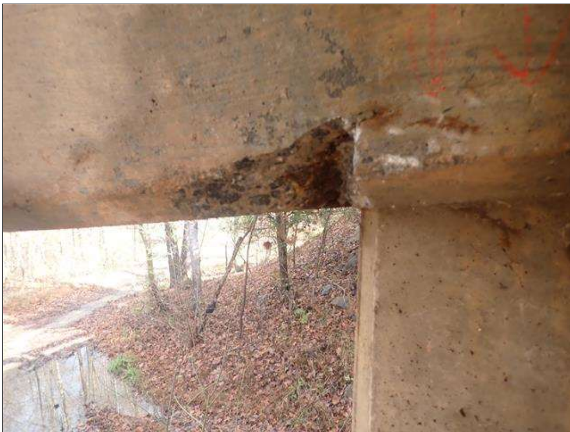
Bent 4 Cap 1: WEST FACE UNDER BEAM 1, SPALL (7IN X 4IN X1-1/2IN) WITH EXPOSED RUSTED REBAR
