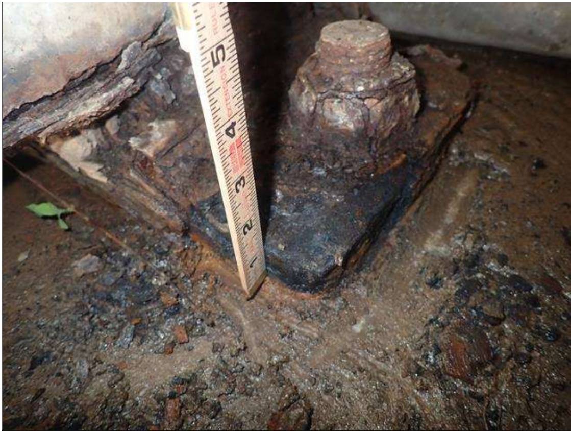
Span 1 Beam 4 - Near Bearing: RUST SCALE WITH SECTION LOSS (UP TO 1/8IN)
