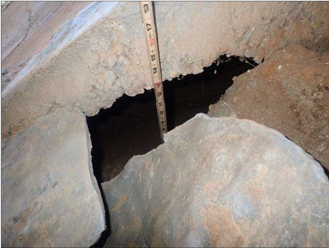
Slope Protection: end bent 1 slope protection under beam 4, failed repair with erosion causing undermining (up to 2ft x up to 1ft deep x full width) of the slope at top and below intermediate diaphragm (photo 1 of 2).
