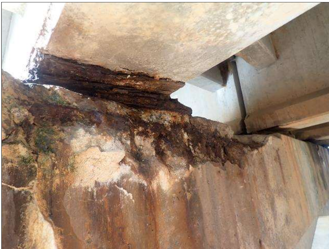
Bent 3 Cap 1: (PAR) 7FT X 12 INCHES X 2 INCHES DEEP SPALL WITH EXPOSED REBAR WITH 15 INCHES X 1 INCHES LOSS OF BEARING ON EAST FACE UNDER BEAM 4
