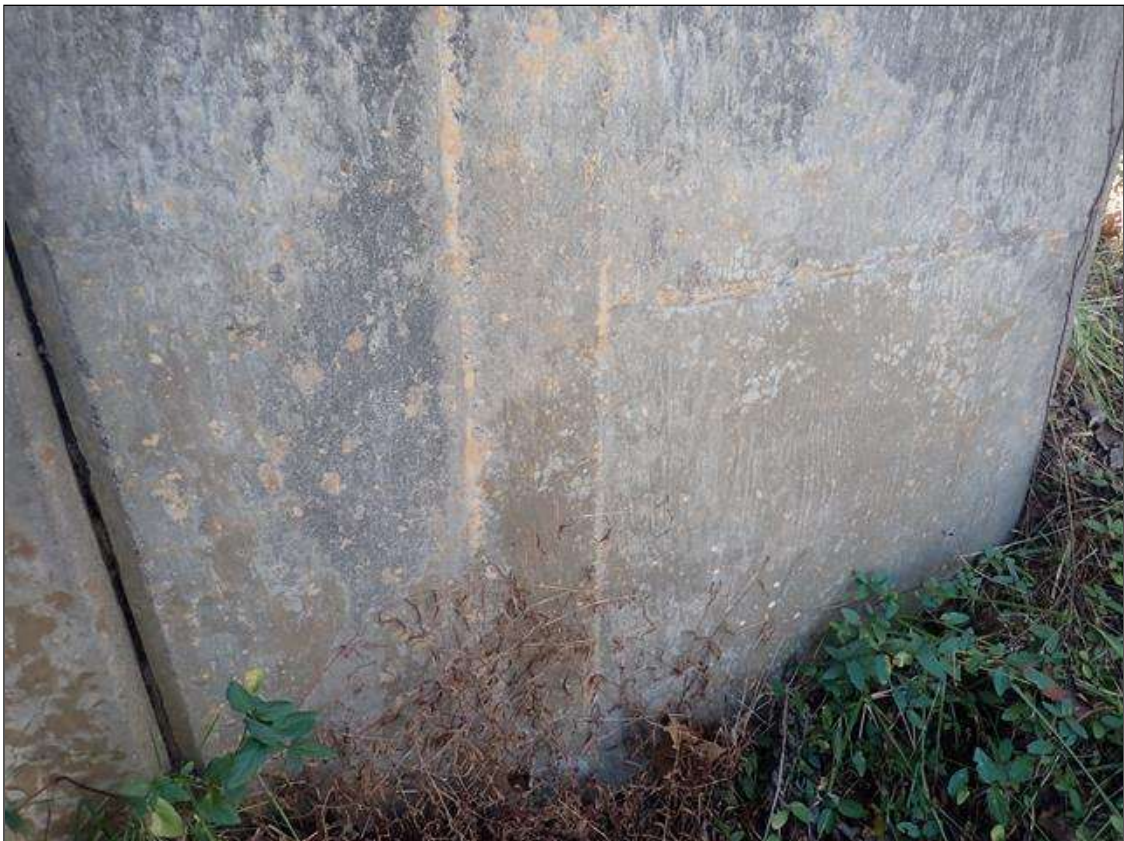
Wingwalls: southwest wingwall, map cracking (full width x up to full height x hairline) with efflorescence
