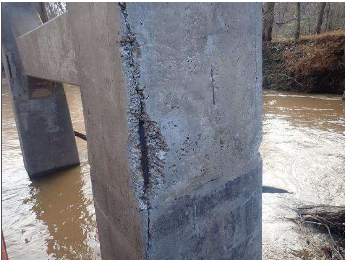
Bent 2 Pile 1: (PAR) 30 INCHES X 10 INCHES X 3 INCHES DEEP SPALL WITH EXPOSED REBAR ON NORTHEAST CORNER
