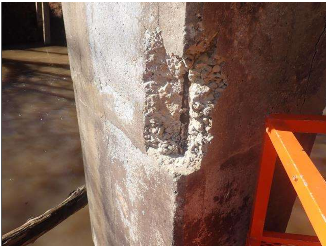
Bent 2 Pile 2: (PAR) 18 INCHES X 12 INCHES X 3 INCHES DEEP SPALL WITH EXPOSED REBAR ON SOUTHEAST CORNER
