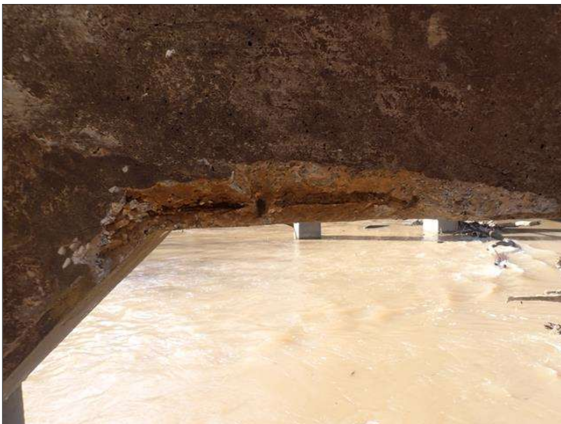
Bent 3 Pile 2: UNDERSIDE OF STRUT NEXT TO PILE 2, SPALL (3FT X 5IN X 3IN) WITH EXPOSED RUSTED REBAR
