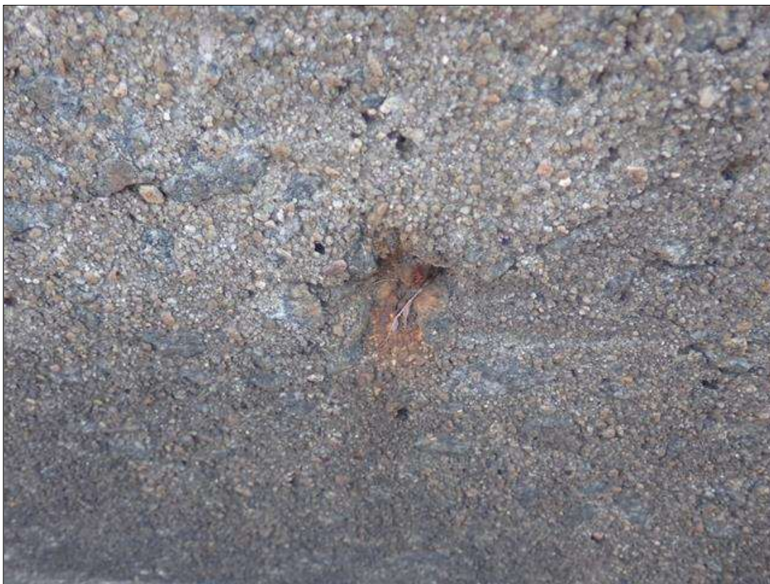
Span 1 Right Bridge Rail: 1 INCHES X 1 INCHES X 1/2 INCHES DEEP SPALL WITH EXPOSED REBAR ON CURB AT POST 4
