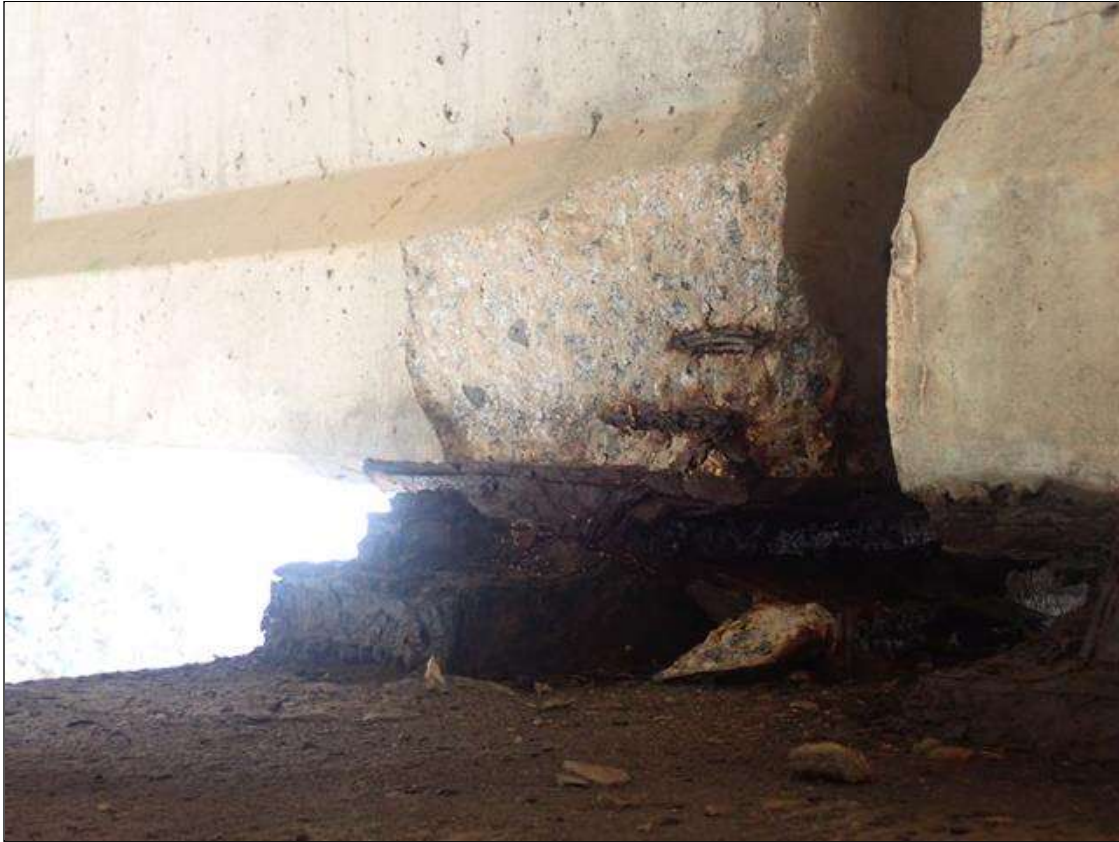
Span 1 Beam 2: (PAR) 12 INCHES X 9 INCHES X 2 INCHES DEEP SPALL WITH EXPOSED PRESTRESSING STRANDS ON RIGHT SIDE OF BOTTOM FLANGE AT BENT 1
