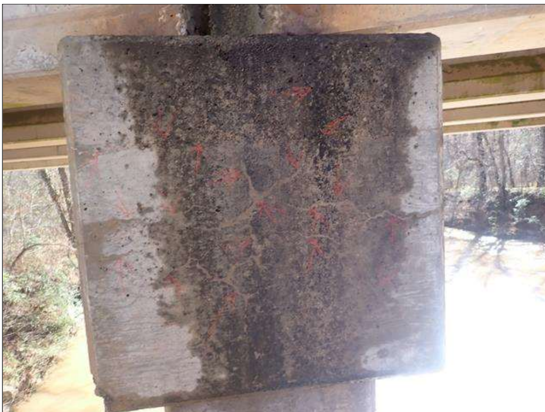
Bent 3 Cap 1: NORTH FACE, MAP CRACKING (FULL WIDTH X FULL HEIGHT X HAIRLINE) WITH EFFLORESCENCE
