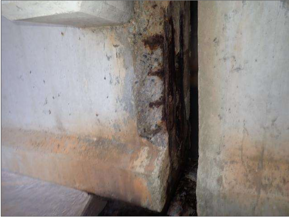
Span 2 Beam 1: (PAR) 16 INCHES X 28 INCHES X 6 INCHES DEEP SPALL WITH EXPOSED PRESTRESSING STRANDS ON BEAM END AT BENT 1
