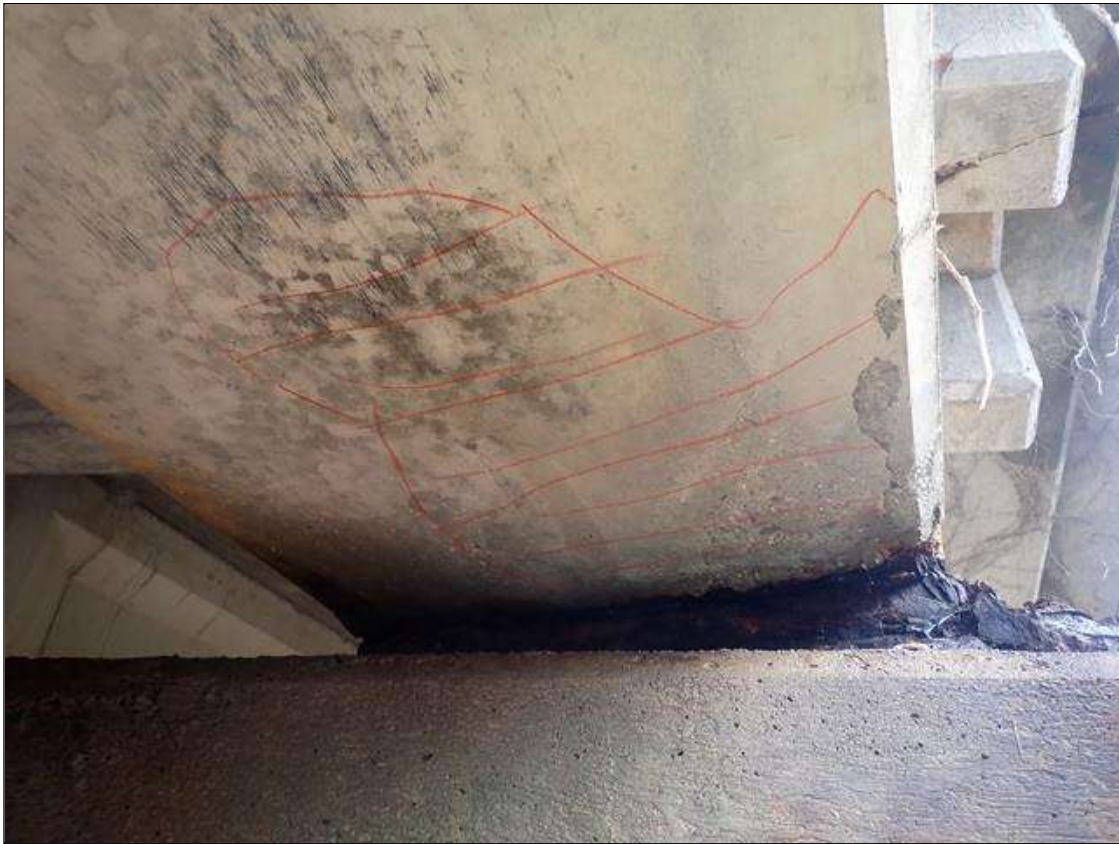
Span 4 Beam 4: 20 INCHES X 14 INCHES AREA OF DELAMINATION ON BOTTOM OF BEAM AT BENT 4
