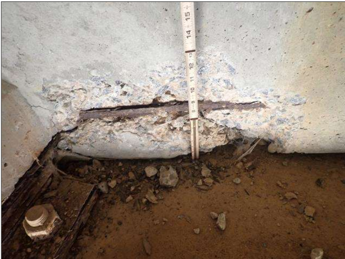
End Bent 1 Abutment: 21 INCHES X 13 INCHES X UP TO 2IN AREA OF SPALLING WITH EXPOSED RUSTED REBAR DEBONDED FROM COBCRETE IN BAY 3 ADJACENT TO BEAM 3
