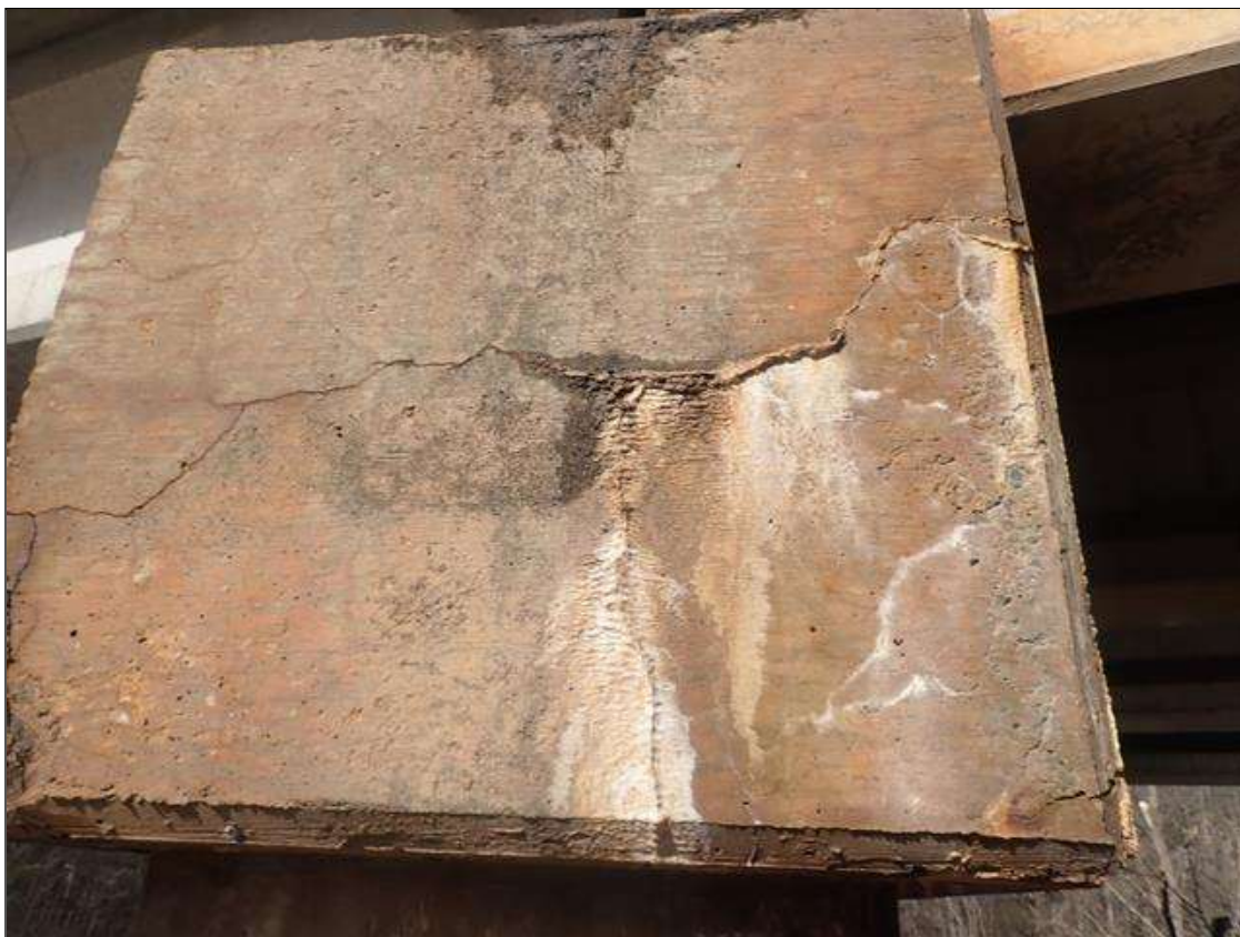
Bent 3 Cap 1: FULL HEIGHT X FULL WIDTH AREA OF VERTICAL (16IN X 1/32IN) AND HORIZONTAL (FULL WIDTH X 1/32IN) CRACKS WITH EFFLORESCENCE ON SOUTH FACE
