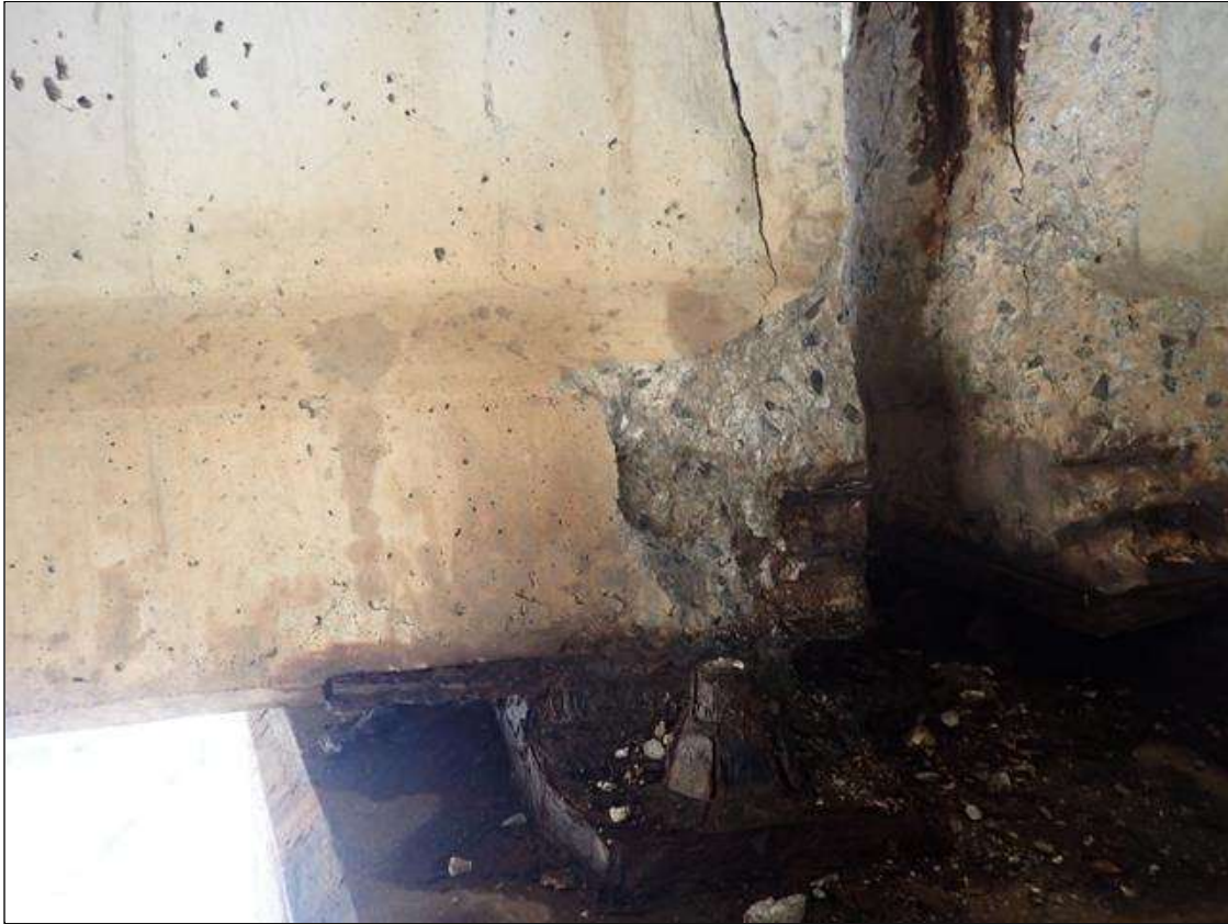
Span 2 Beam 3: (PAR) 10 INCHES X 10 INCHES X 2 1/2 INCHES DEEP SPALL WITH EXPOSED PRESTRESSING STRANDS ON LEFT SIDE OF BOTTOM FLANGE AT BENT 1
