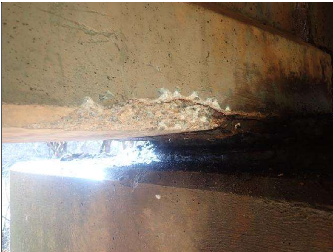
Span 5 Beam 4: BOTTOM FLANGE NORTH FACE AT BENT 4, SPALL (11IN X 3IN X 1-1/2IN)
