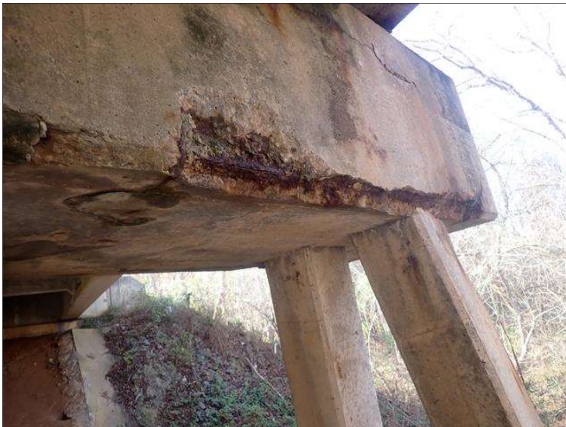
Bent 1 Cap 1: (PAR) 7 FEET X 9 INCHES X 3 INCHES DEEP SPALL WITH EXPOSED REBAR AND AREA OF DELAMINATION ON EAST FACE BETWEEN PILES 1 AND 2
