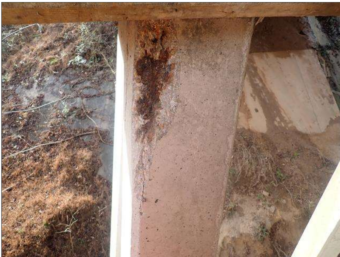
Bent 1 Row 2 Pile 5: (PAR) 18 INCHES X 5 INCHES X 3 INCHES DEEP SPALL WITH EXPOSED STRAND ON SOUTHEAST CORNER
