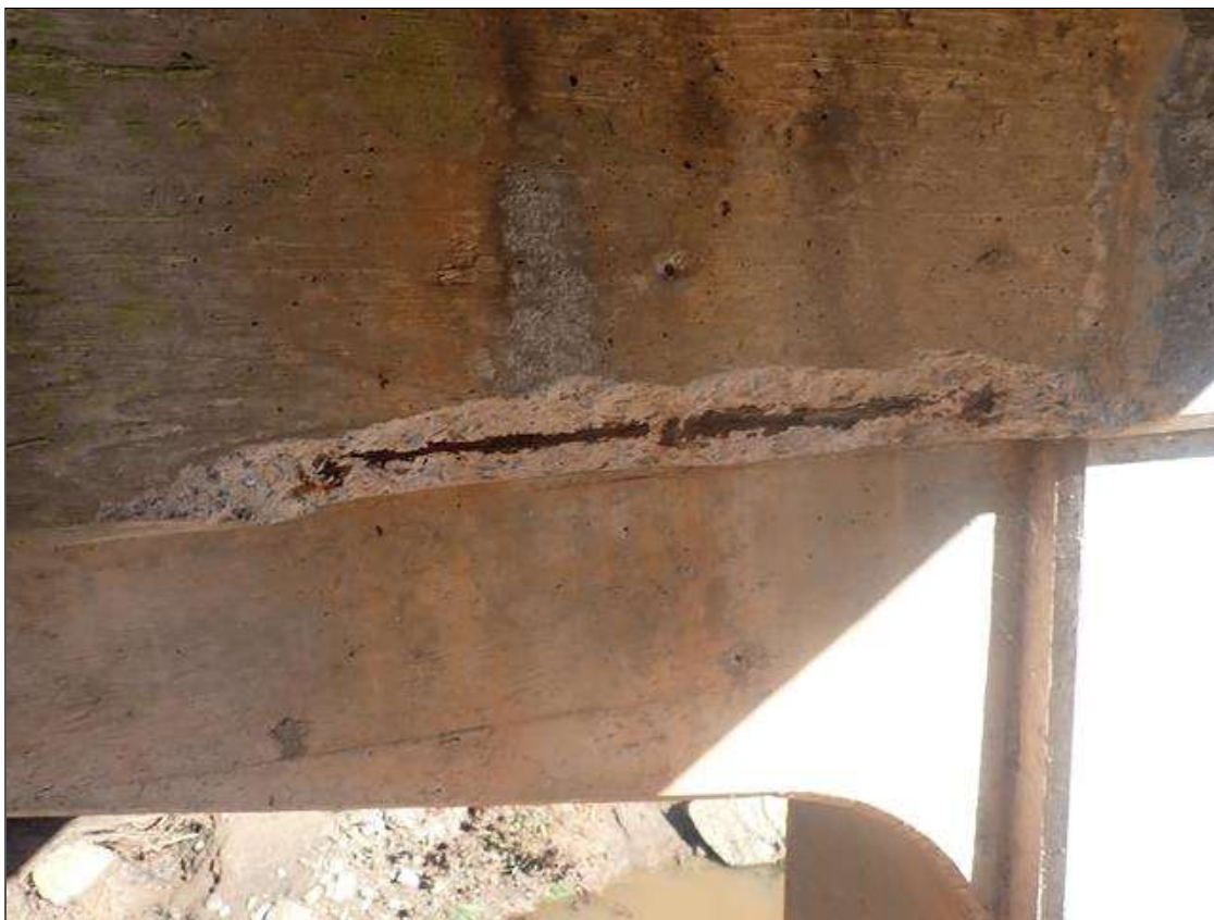
Bent 3 Cap 1: (PAR) 53 INCHES X 7 INCHES X 3 INCHES DEEP SPALL WITH EXPOSED REBAR ON WEST FACE UNDER BAY 3
