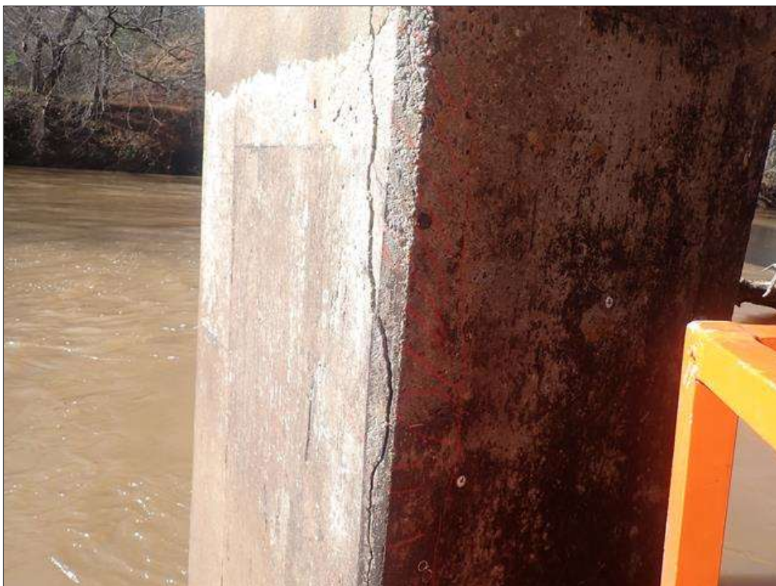
Bent 3 Pile 2: (PAR) 10 FEET X 8 INCHES X 2 INCHES DEEP SPALL/DELAMINATION WITH EXPOSED REBAR ON SOUTHEAST CORNER (PHOTO 1 OF 2)
