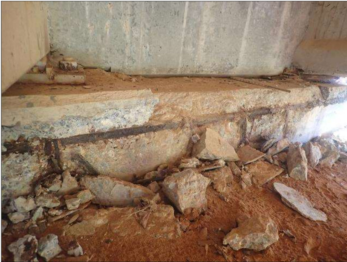
End Bent 2 Cap 1: (PAR) 9 FEET X 14 INCHES X 5 INCHES DEEP SPALL WITH EXPOSED REBAR AND AREA OF DELAMINATION UNDER BAY 3
