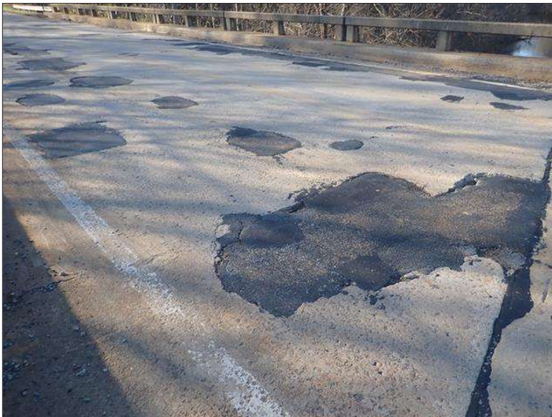
Span 2 Deck: both lanes scattered throughout, patched areas (up to 31ft x 4ft)
