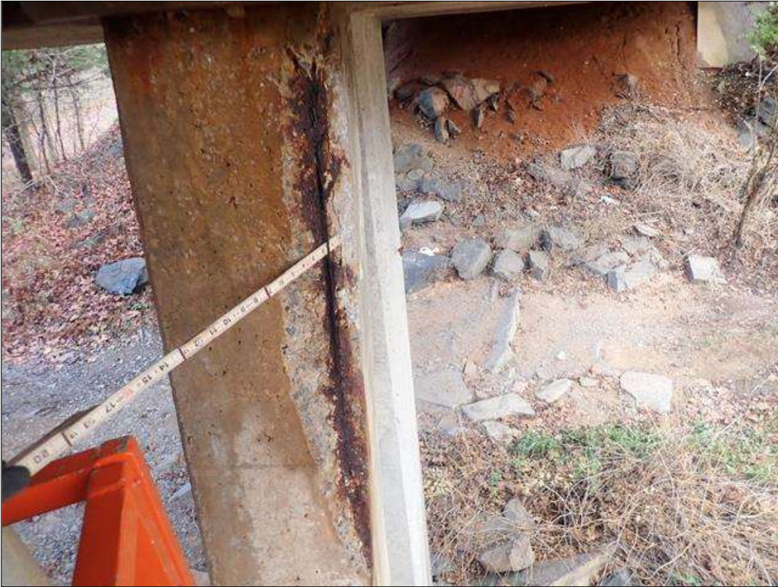
Bent 4 Row 1 Pile 4: (PAR) 36 INCHES X 6 INCHES X 2 INCHES DEEP SPALL WITH EXPOSED STRAND (UP TO 90% LOSS ON STRAND) ON SOUTHWEST CORNER
