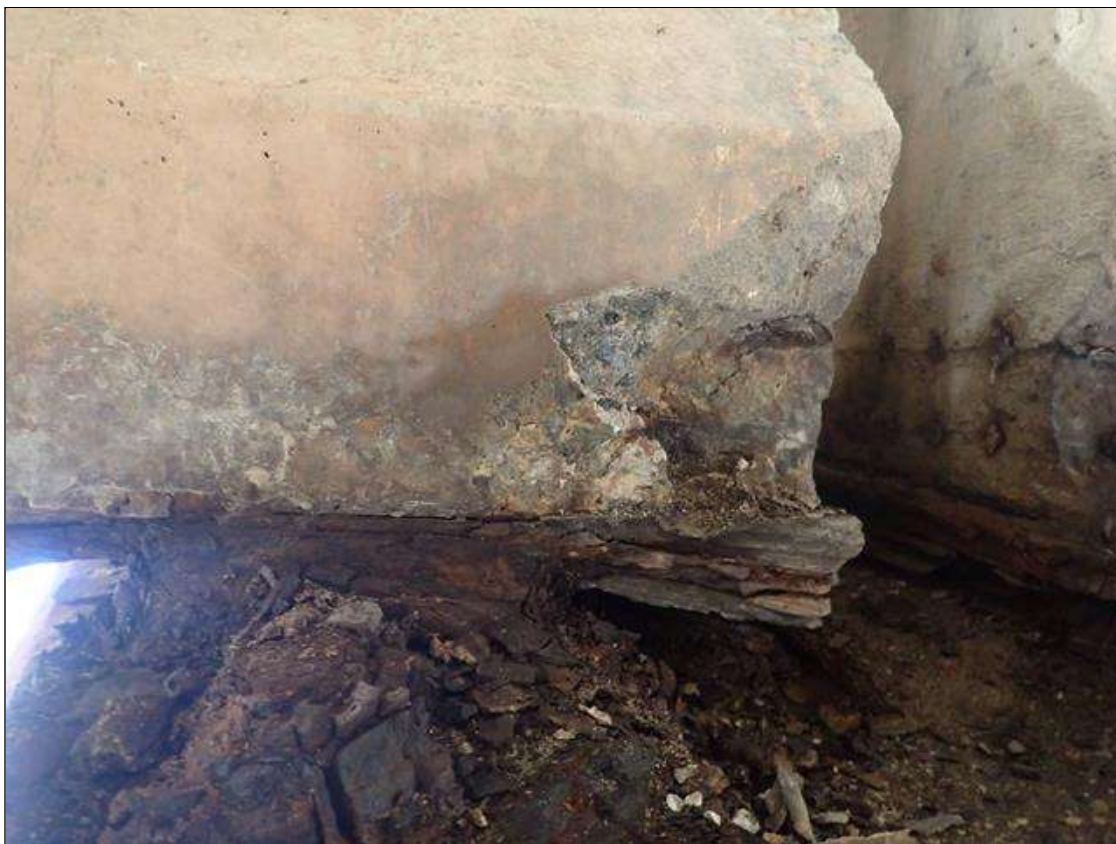
Span 2 Beam 3: (PAR) 8 INCHES X 7 INCHES X 2 1/2 INCHES DEEP SPALL WITH EXPOSED PRESTRESSING STRANDS ON RIGHT SIDE OF BOTTOM FLANGE AT BENT 2
