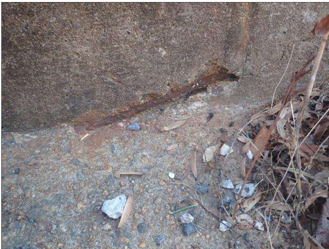
Span 1 Left Bridge Rail: END POST EAST FACE AT END BENT 1, SPALL (6IN X 4IN X 1-1/2IN) WITH EXPOSED RUSTED REBAR
