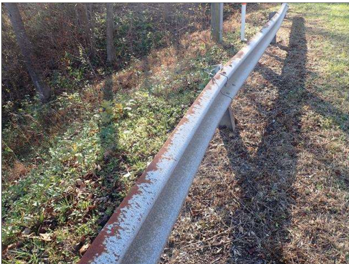
General Comments and Misc Items: southwest guardrail at 25ft from end bent 1, impact damage (12ft)
