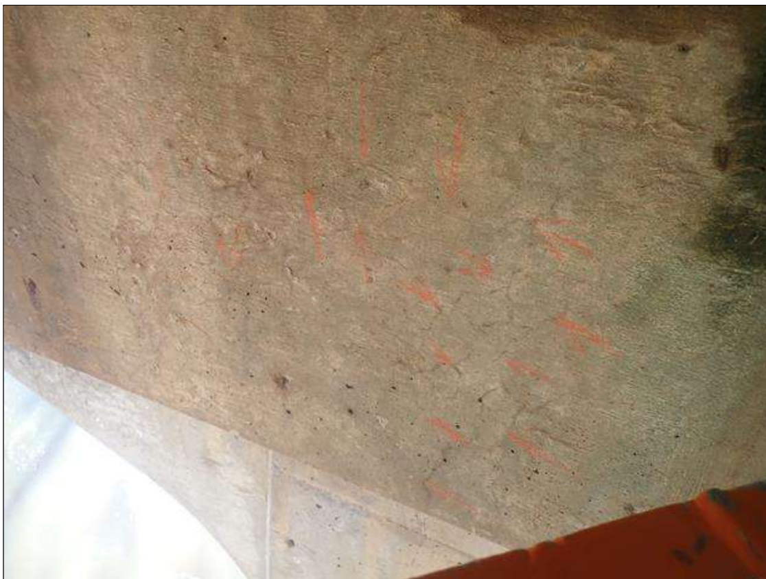
Bent 2 Cap 1: EAST FACE SCATTERED THROUGHOUT, MAP CRACKING (FULL HEIGHT X UP TO 4FT X HAIRLINE)
