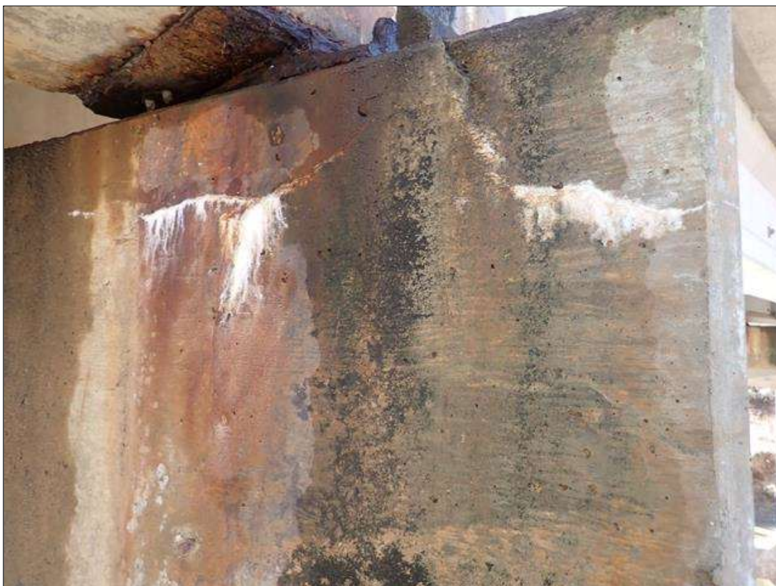
Bent 3 Cap 1: 3 FEET X 3 FEET AREA OF HAIRLINE VERTICAL AND HORIZONTAL CRACKS UP TO 1/32IN WITH EFFLORESCENCE ON EAST FACE AT NORTH END
