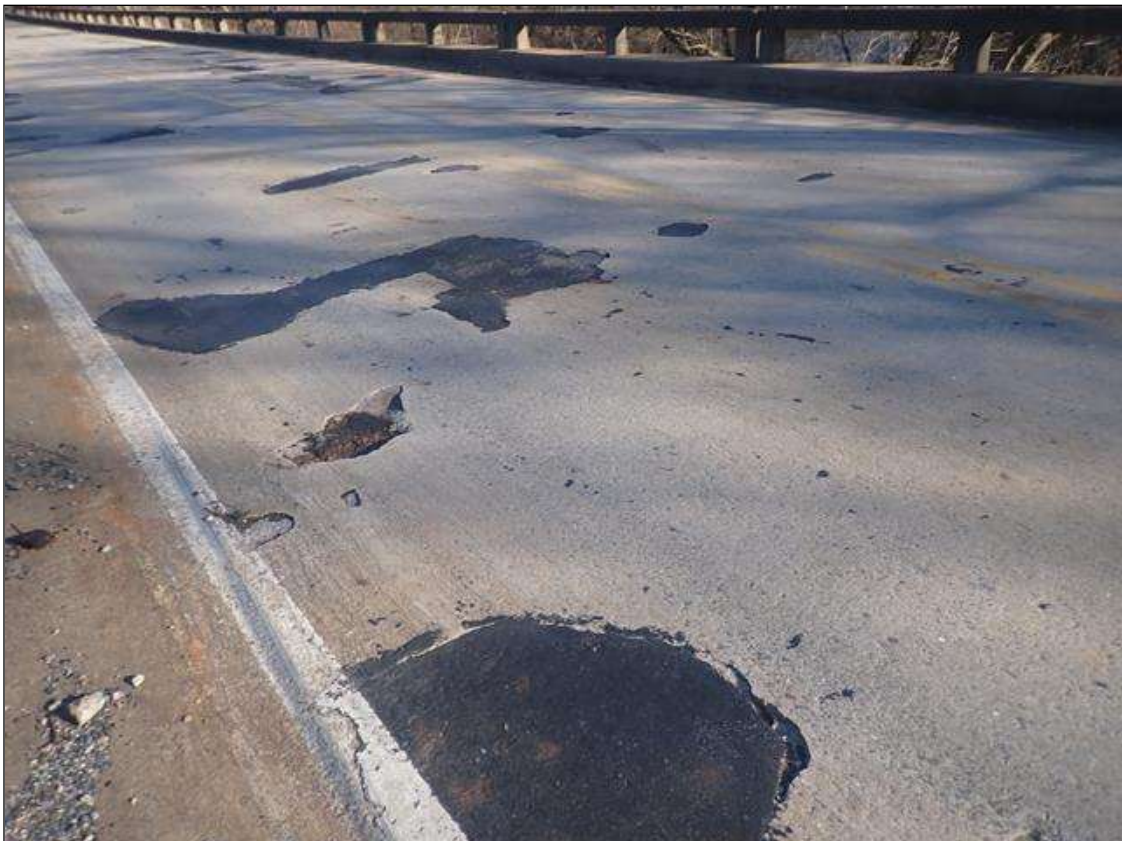
Span 1 Deck: both lanes scattered throughout, patched areas (up to 7ft x 4ft)
