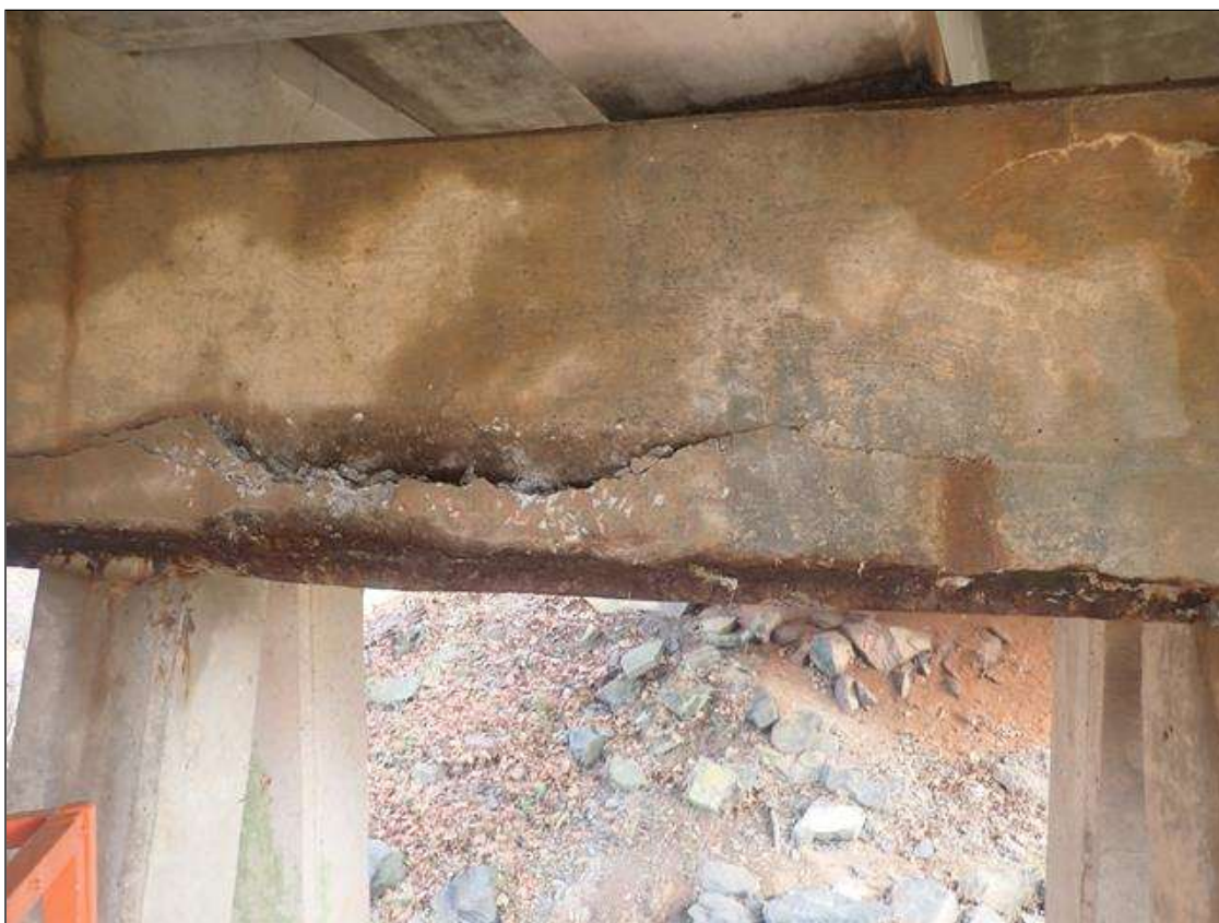
Bent 4 Cap 1: (PAR) WEST FACE UNDER BEAM 3, SPALL/DELAMINATION (95IN X 12IN X UP TO 2-1/2IN) WITH EXPOSED RUSTED REBAR
