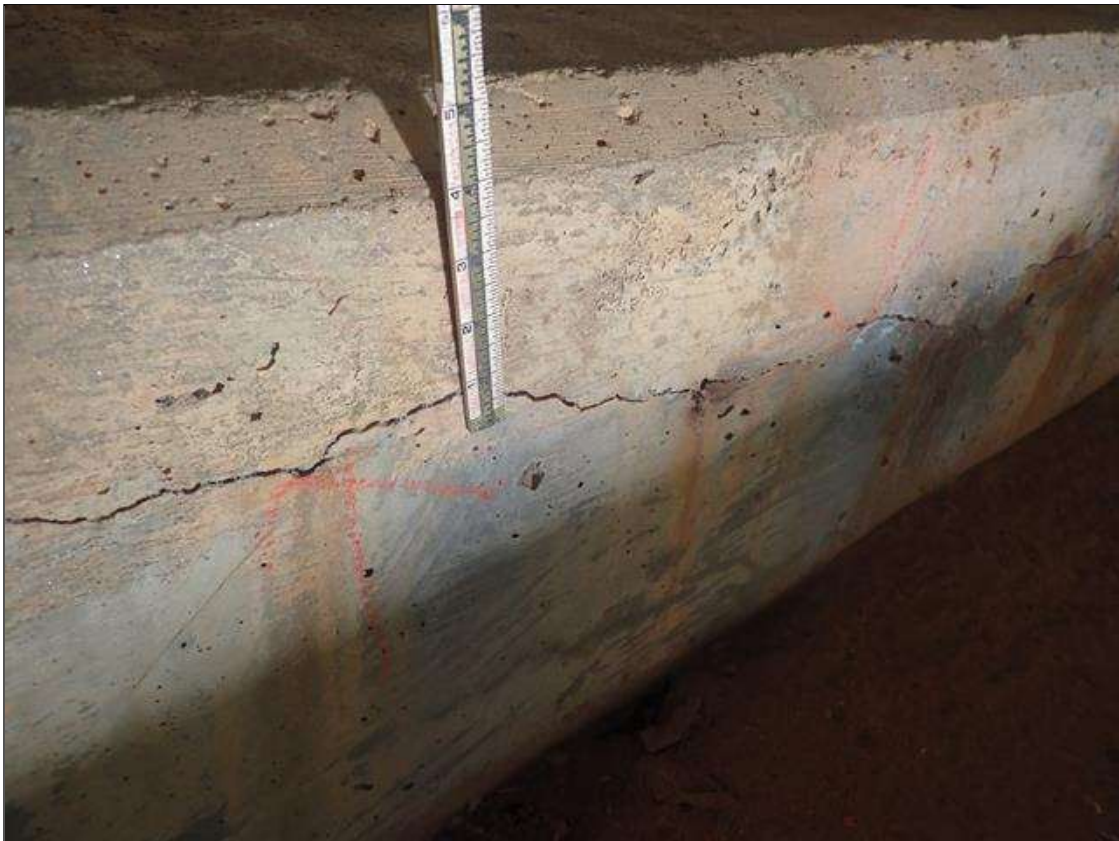
End Bent 2 Cap 1: 5 FEET UP TO 1/8 INCHES HORIZONTAL CRACK WITH RUST STAINS UNDER BAYS 1 AND 2
