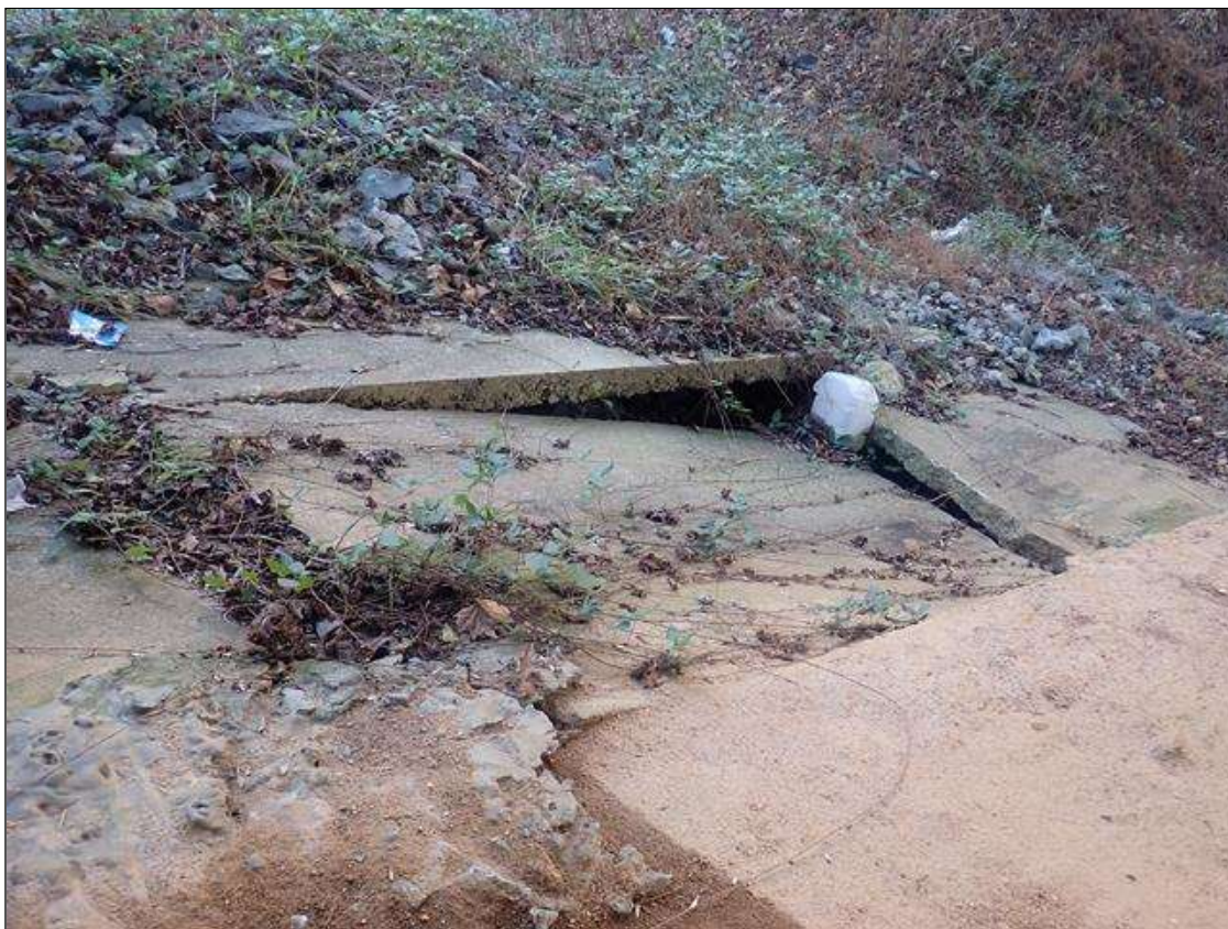
Slope Protection: end bent 1 slope protection north end at base, broken concrete and separation of slope allowing erosion with undermining (6ft x up to 1ft deep x full width) of the slope
