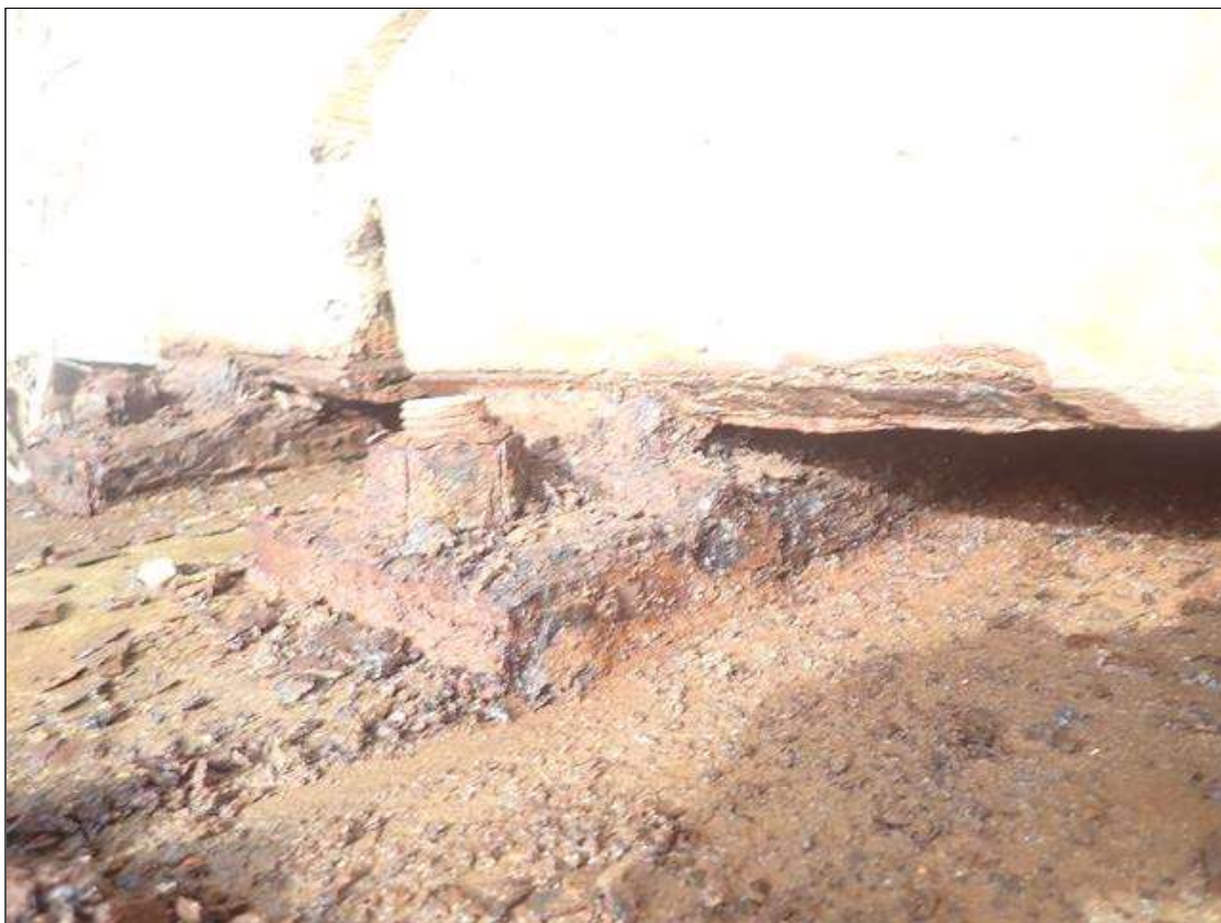
Span 5 Beam 4 - Near Bearing: RUST SCALE WITH SECTION LOSS (UP TO 1/8IN LOSS)
