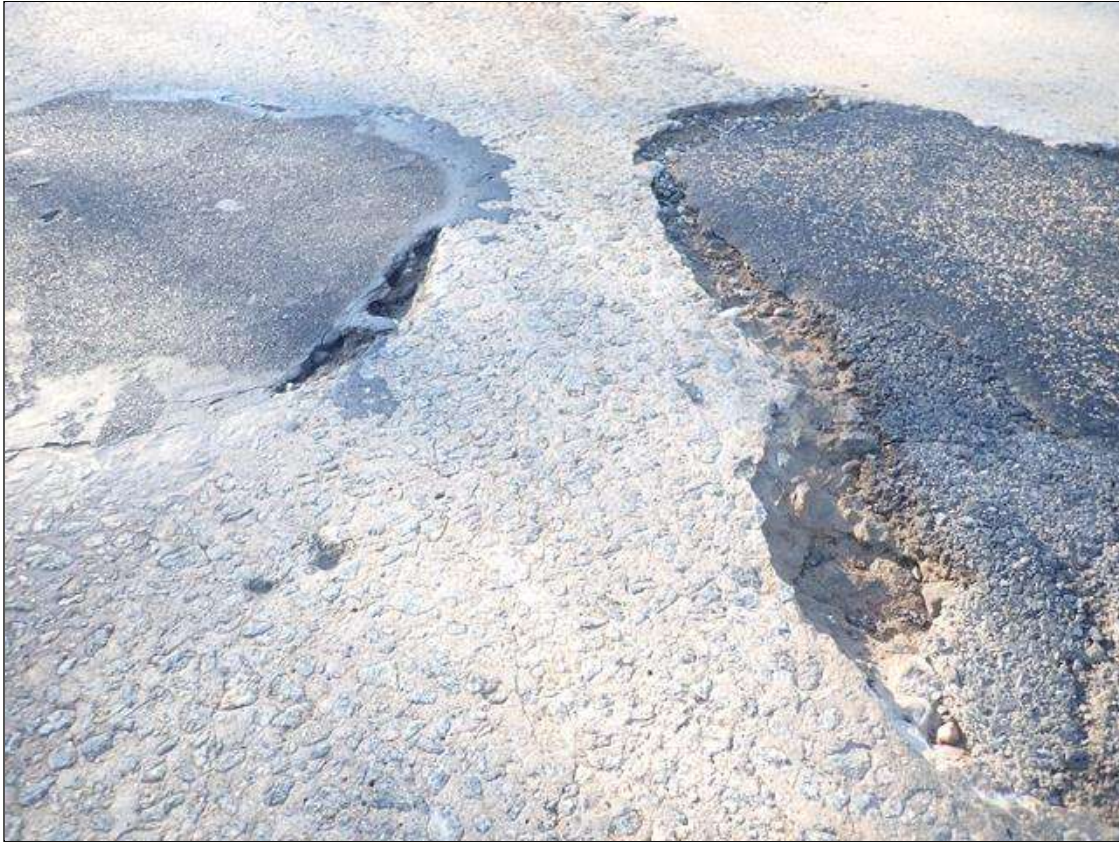
Span 2 Deck: both lanes scattered throughout, spalls (up to 3ft x up to 12in x 1in) mainly at edges of previously patched areas (photo 2 of 2)
