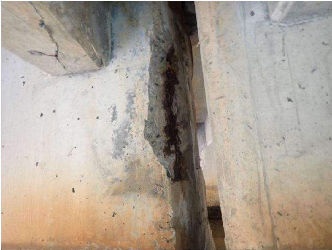
Span 2 Beam 2: (PAR) 24 INCHES X 16 INCHES X 4 INCHES DEEP SPALL WITH EXPOSED PRESTRESSING STRANDS ON BEAM END AT BENT 1
