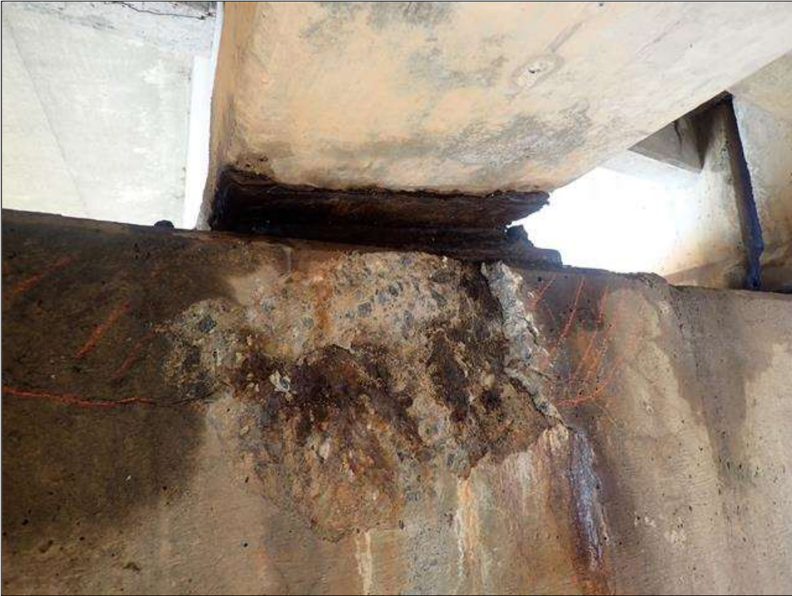
Bent 3 Cap 1: (PAR) 40 INCHES X 16 INCHES X 2 INCHES DEEP SPALL WITH EXPOSED REBAR AND AREA OF DELAMINATION ON EAST FACE UNDER BEAM 2
