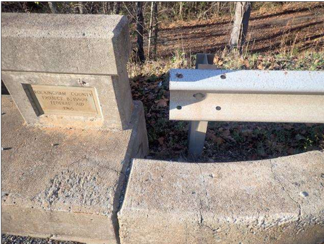
General Comments and Misc Items: northeast guardrail not attached to bridge rail
