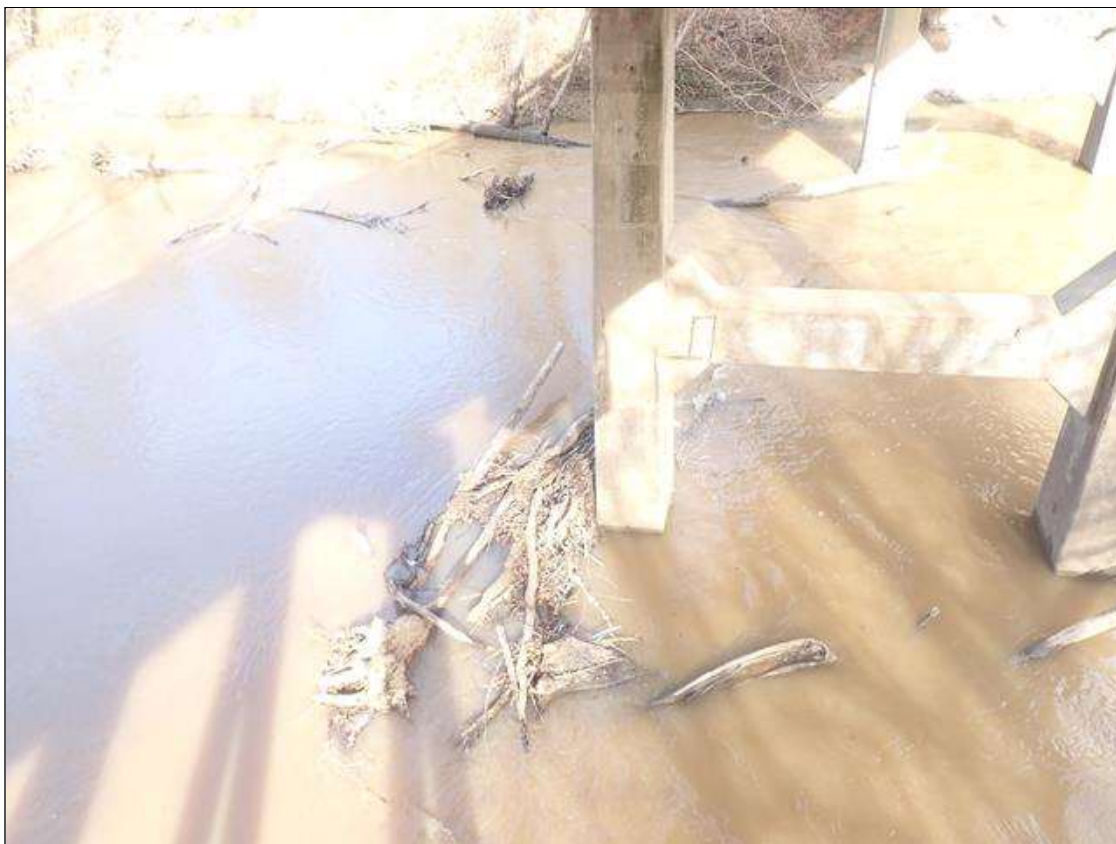
Drift: upstream at bent 2 pile 1, drift accumulation (2cy)
