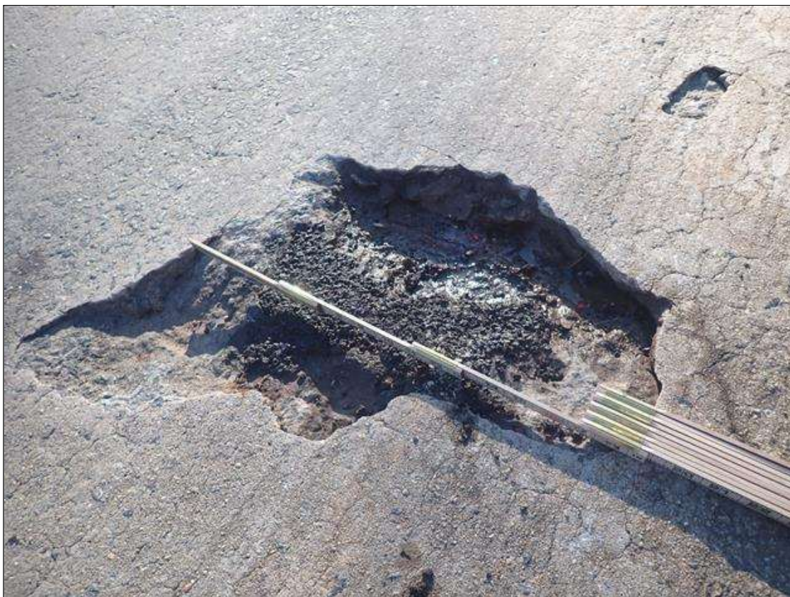
Span 1 Deck: (PAR) westbound lane at midspan, spall (2ft x up to 16in x 2in) with exposed rusted rebar
