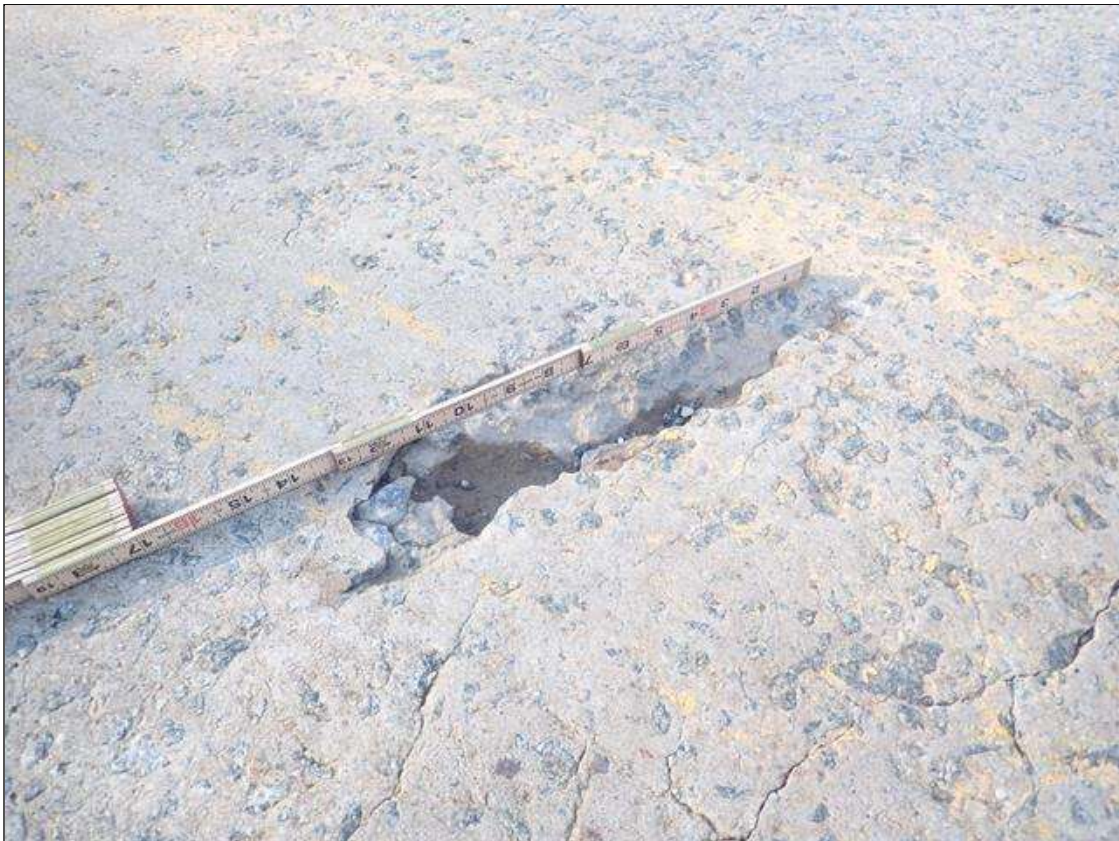
Span 2 Deck: both lanes scattered throughout, spalls (up to 3ft x up to 12in x 1in) mainly at edges of previously patched areas (photo 1 of 2)
