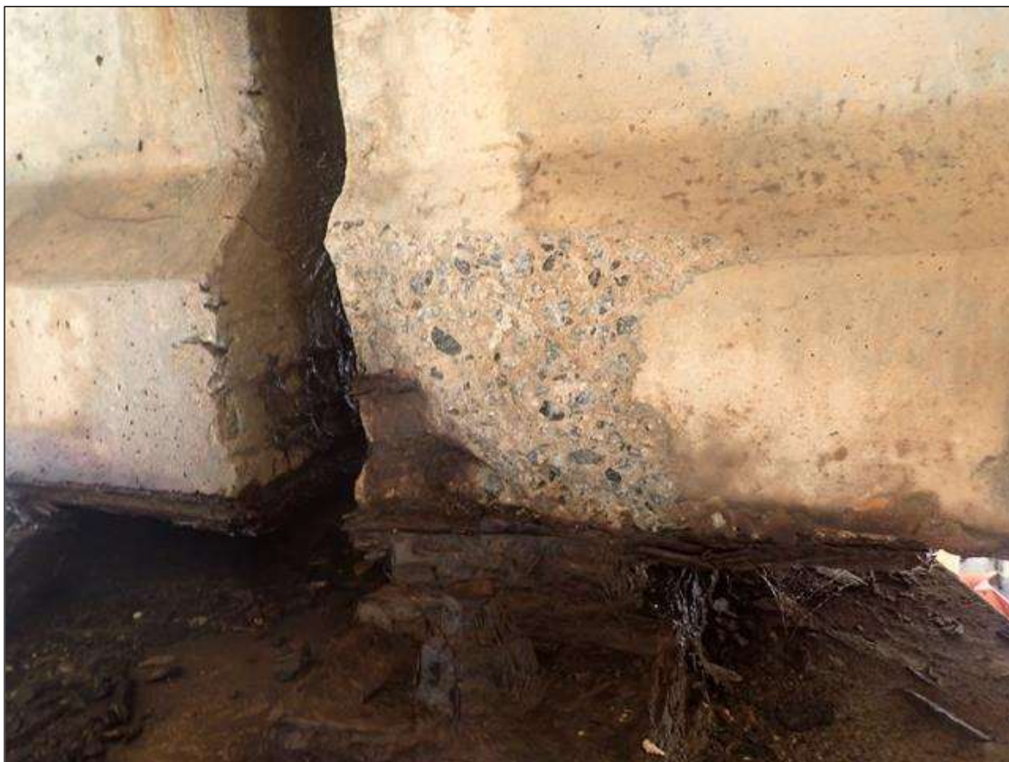
Span 5 Beam 3: (PAR) 18 INCHES X 8 INCHES X 2 INCHES DEEP SPALL WITH EXPOSED PRESTRESSING STRANDS ON RIGHT SIDE OF BOTTOM FLANGE AT BENT 4
