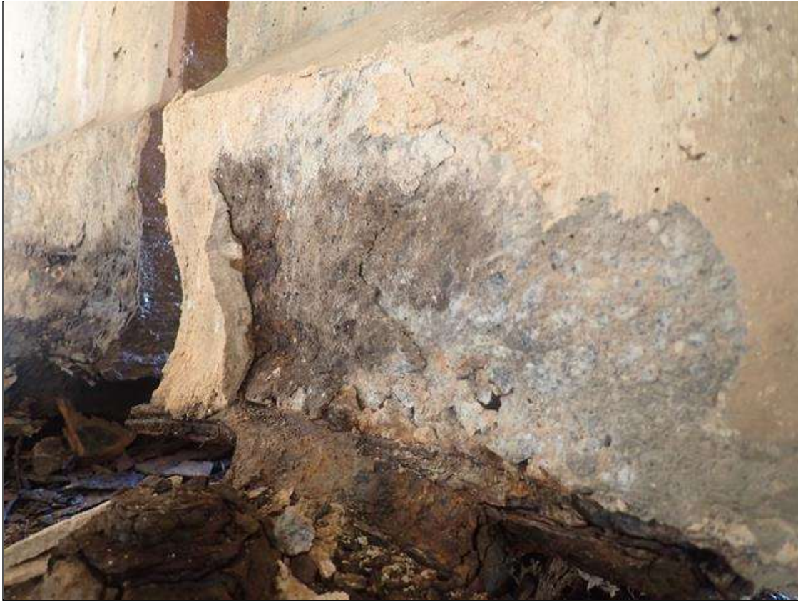
Span 3 Beam 4: (PAR) LEFT SIDE OF BOTTOM FLANGE AT BENT 3, SPALL (17IN X 6IN X UP TO 2IN) WITH EXPOSED RUSTED STRANDS AT FAILED PATCHED AREA
