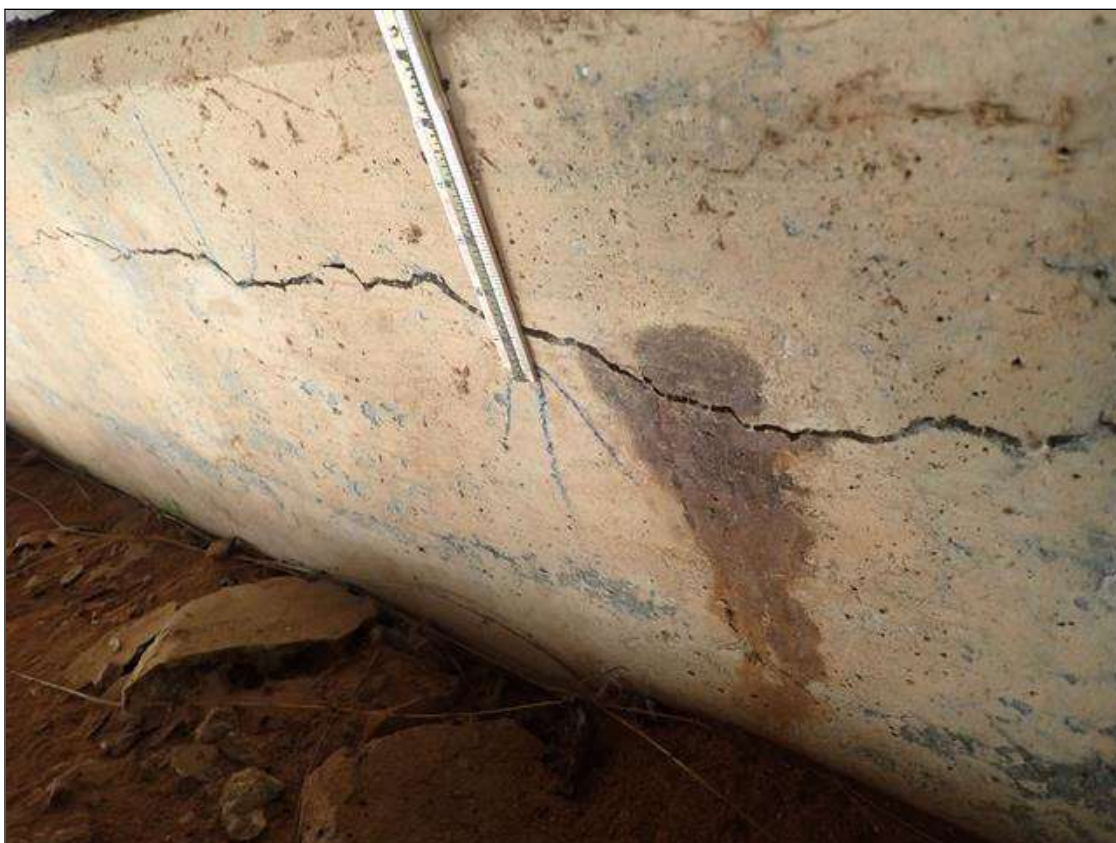
End Bent 1 Cap 1: 60 INCHES UP TO 1/8 INCHES AREA OF HAIRLINE HORIZONTAL CRACK UNDER BAYS 2 AND 3
