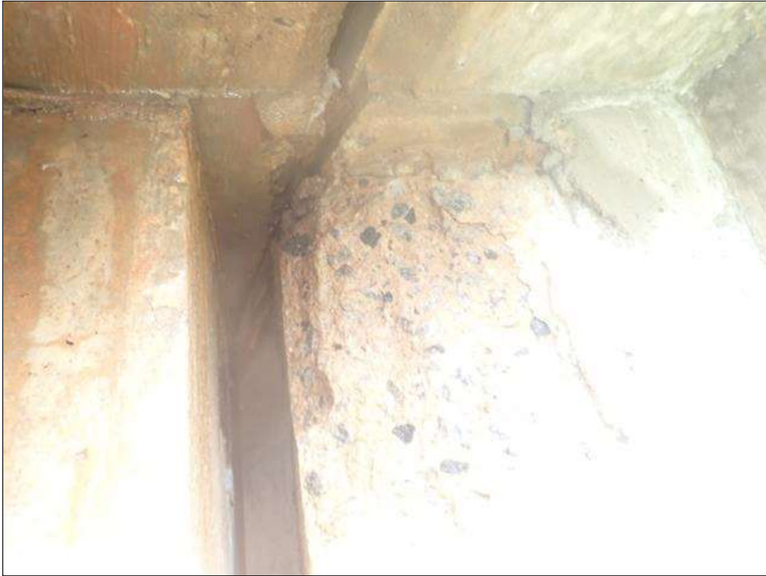
Span 5 Beam 4: 6 INCHES X 36 INCHES X UP TO 1-1/2 INCHES DEEP SPALL ON RIGHT SIDE OF WEB AT BENT 4 (PHOTO 2 OF 2)
