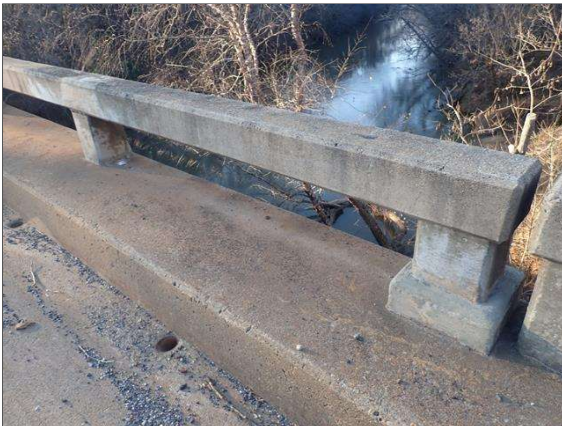
Span 4 Left Bridge Rail: 6 FEET REPLACED RAIL SECTION AT POST 2
