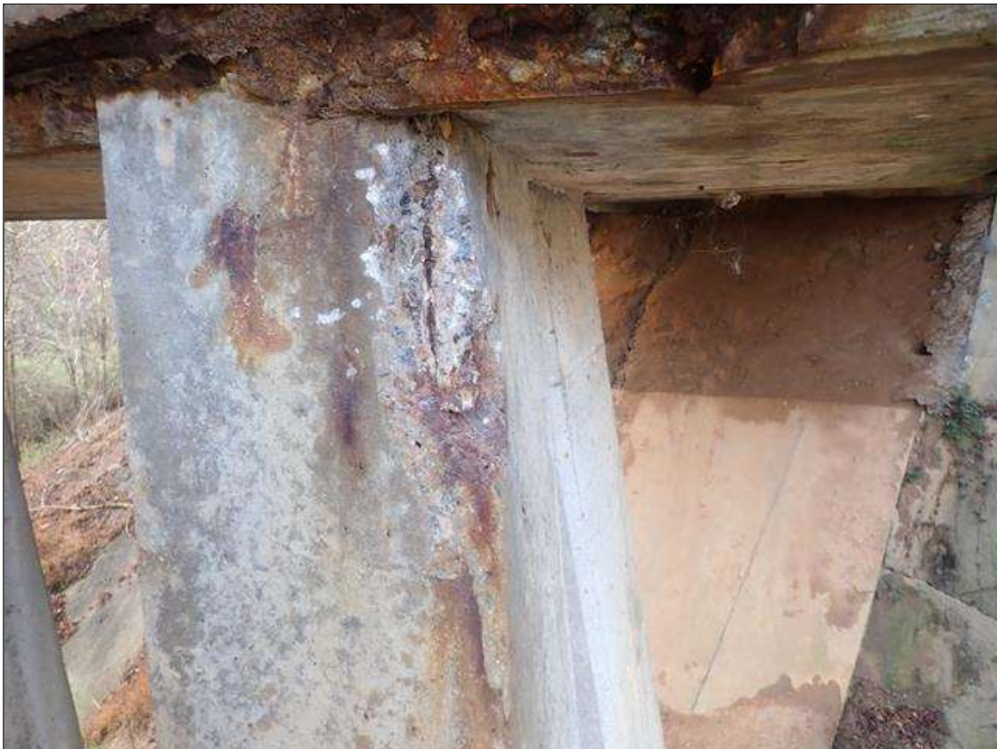
Bent 1 Row 2 Pile 1: (PAR) 16 INCHES X 3 INCHES X 4 INCHES DEEP SPALL WITH EXPOSED STRAND ON NORTHEAST CORNER
