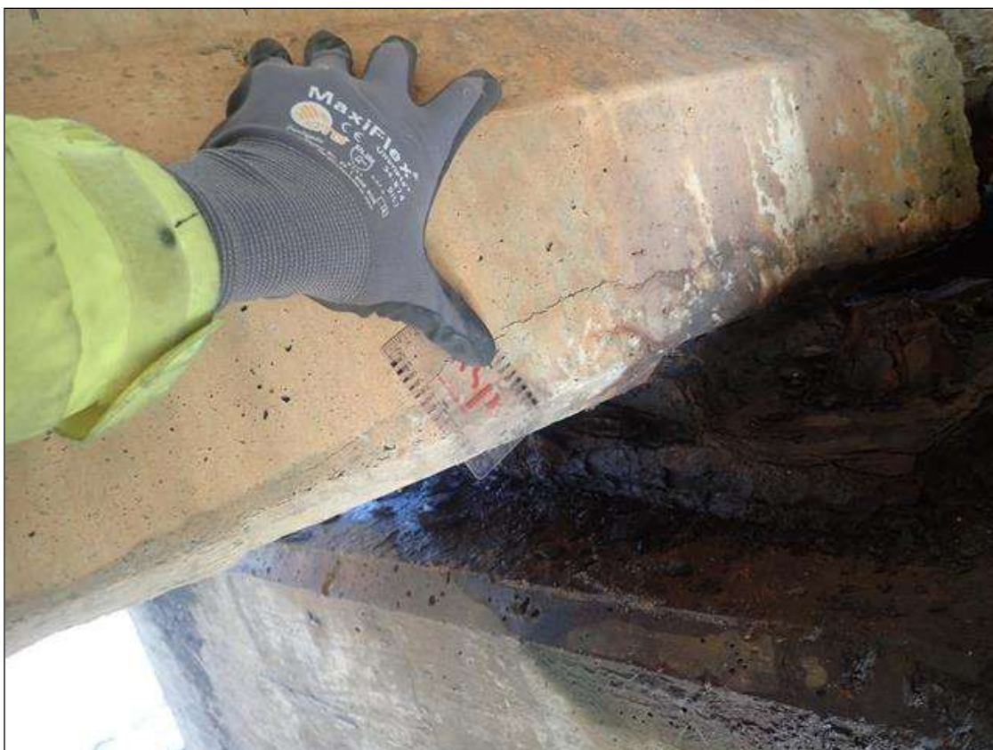
Span 3 Beam 1: BOTTOM FLANGE RIGH SIDE AT BENT 4, HORIZONTAL CRACK (12IN X UP TO 0.016IN)
