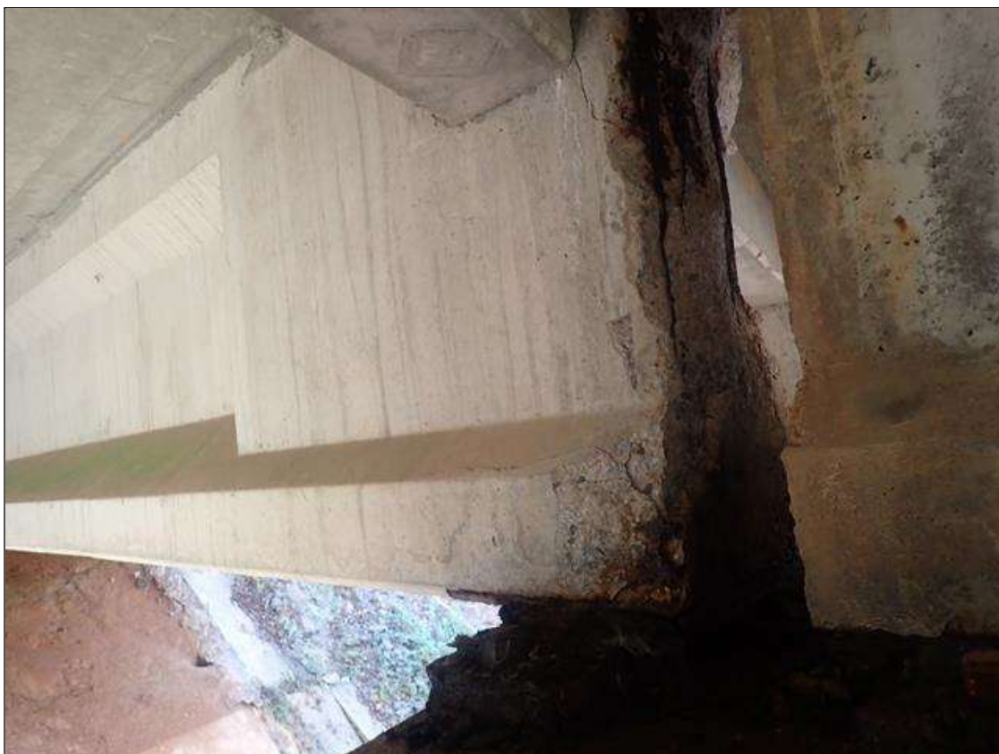
Span 1 Beam 3: (PAR) 16 INCHES X 41 INCHES X 2 INCHES DEEP SPALL WITH EXPOSED PRESTRESSING STRANDS ON BEAM END AT BENT 1
