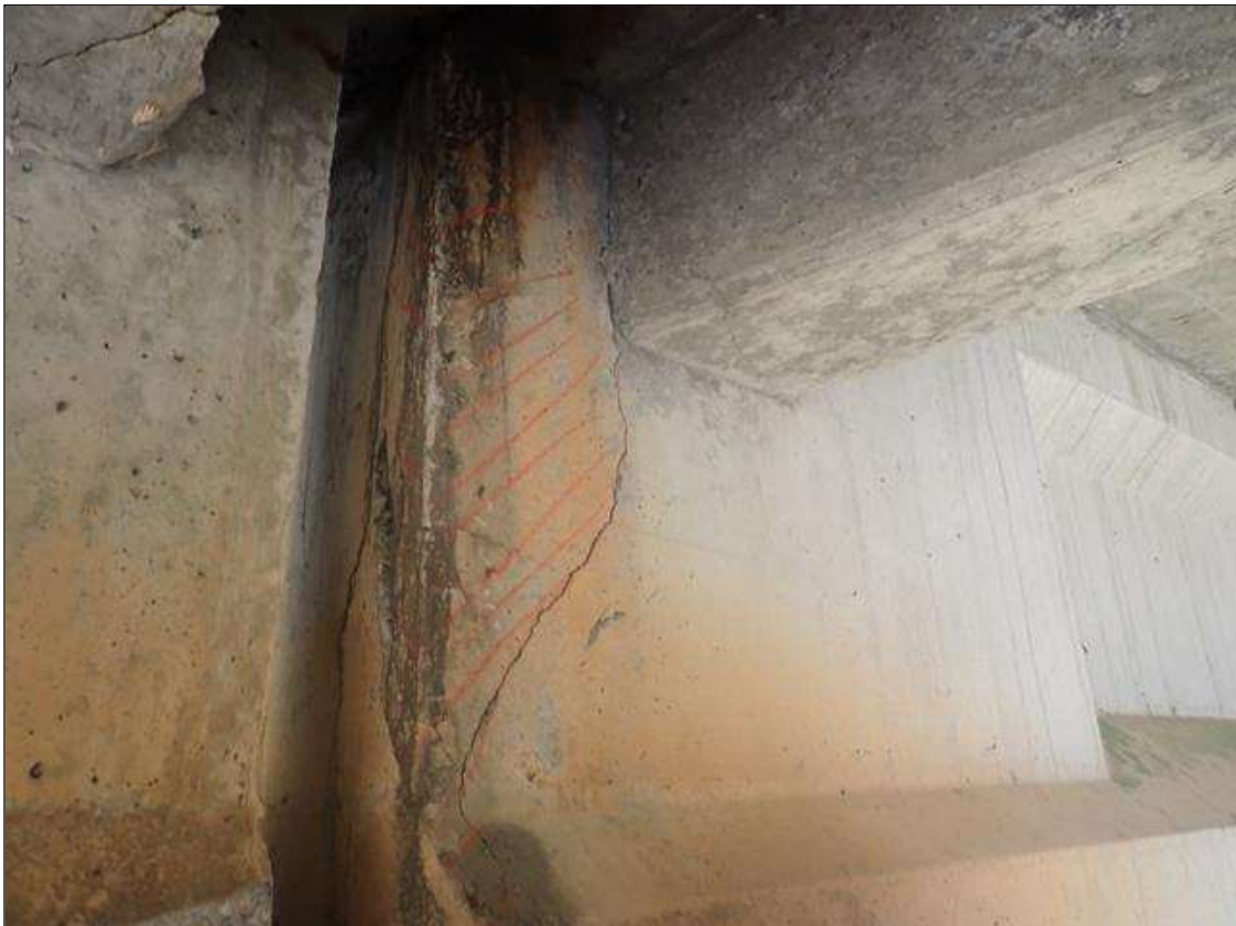
Span 2 Beam 3: 1 FEET X 30 INCHES X 4 INCHES DELAMINATION ON LEFT SIDE OF WEB AT BENT 2
