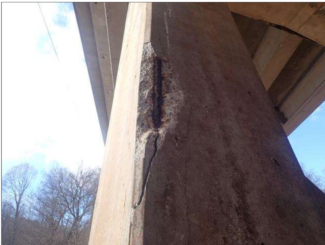
Bent 3 Pile 2: (PAR) 10 FEET X 8 INCHES X 2 INCHES DEEP SPALL/DELAMINATION WITH EXPOSED REBAR ON SOUTHEAST CORNER (PHOTO 2 OF 2)
