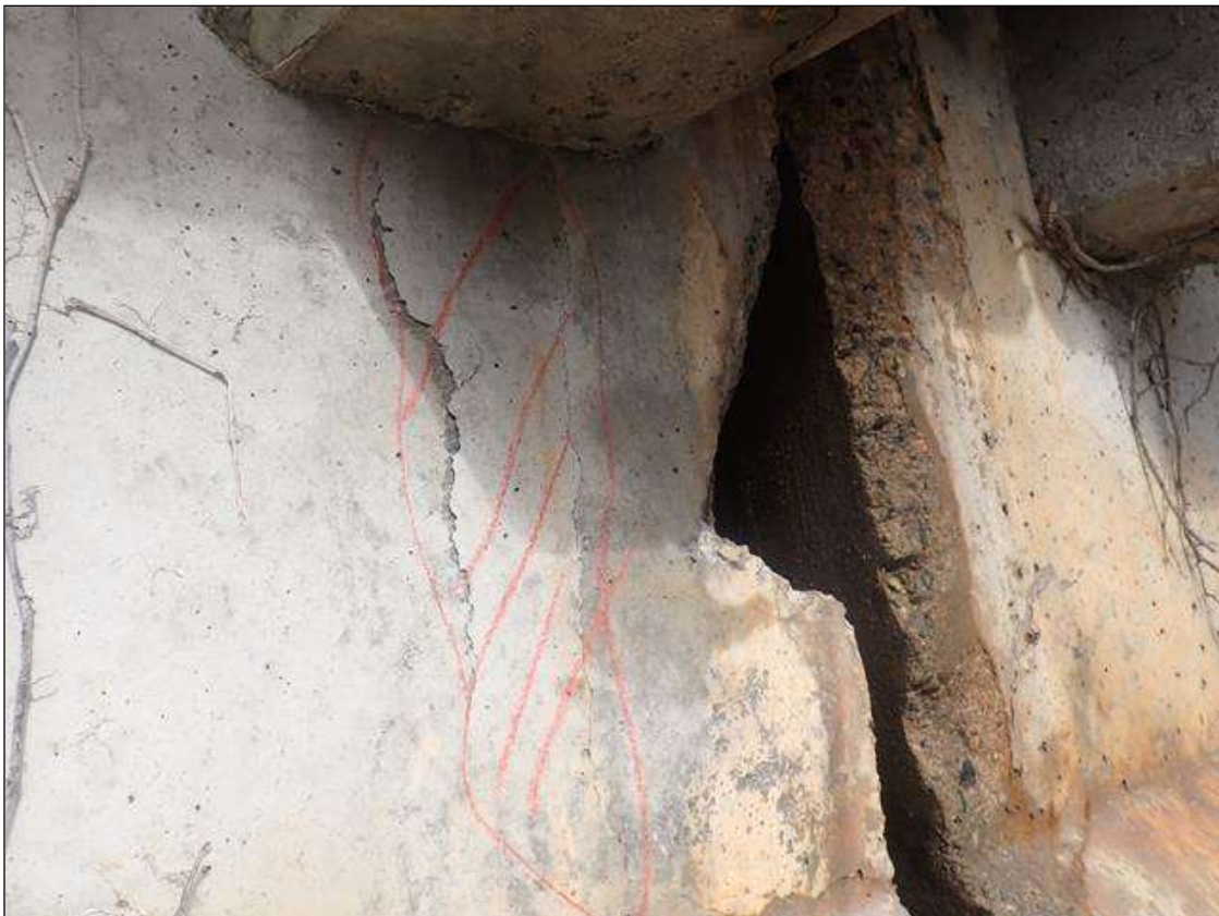
Span 4 Beam 4: EAST END OF WEB AT BENT 4, SPALL (18IN X 12IN X UP TO 3IN) WITH ADJACENT DELAMINATION (22IN X 5IN) ON SOUTH FACE (PHOTO 1 OF 2)
