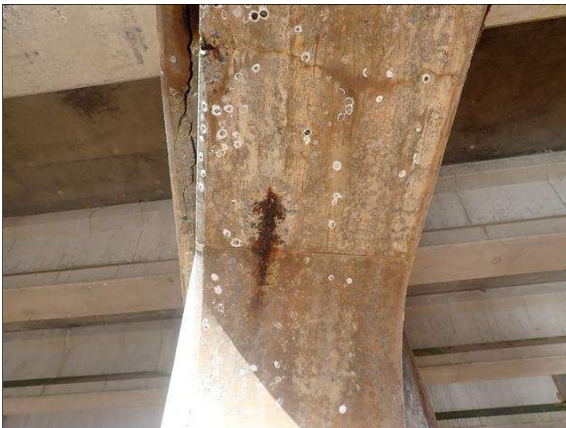
Bent 3 Pile 2: (2) UP TO 12 INCHES X 6 INCHES X 1 INCHES DEEP SPALL WITH EXPOSED REBAR ON BOTTOM OF CORBEL AT SOUTH END
