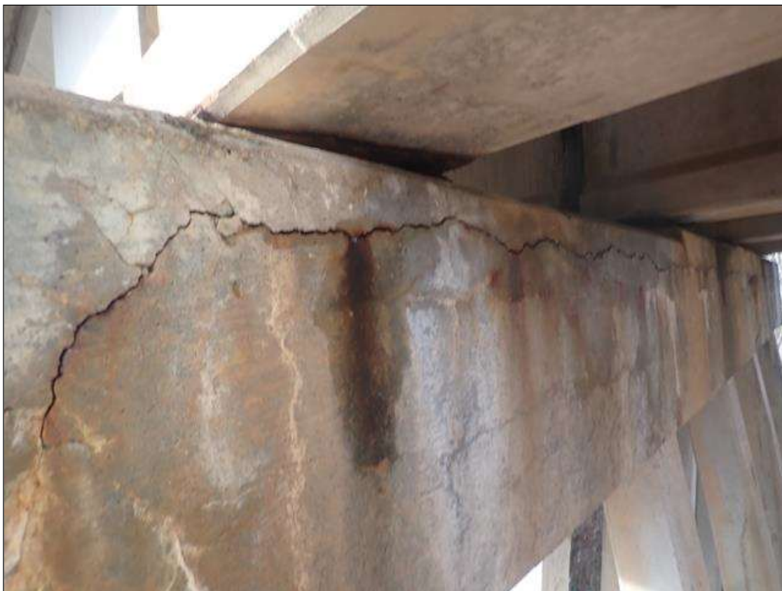
Bent 1 Cap 1: 12 FEET X 1 FEET AREA OF DELAMINATION WITH UP TO 3/16 INCHES HORIZONTAL CRACK WITH EFFLORESCENCE AND RUST STAINS ON EAST FACE AT SOUTH END
