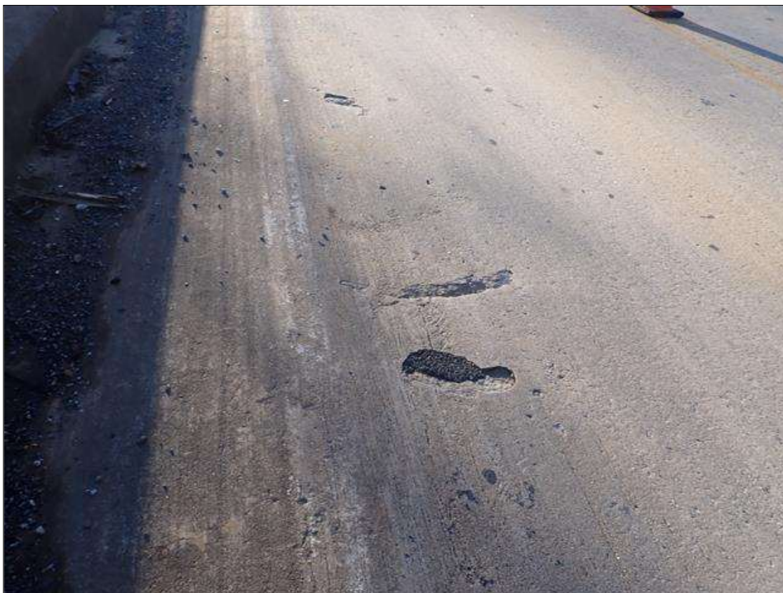
Span 5 Deck: (4) UP TO 18 INCHES X 24 INCHES X 1 INCHES DEEP SPALLS AND AREA OF DELAMINATION SCATTERED THROUGHOUT EASTBOUND LANE
