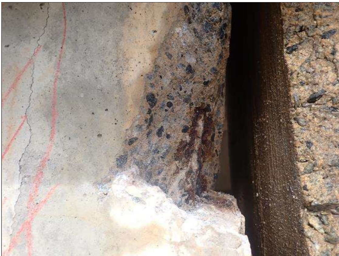
Span 4 Beam 4: EAST END OF WEB AT BENT 4, SPALL (18IN X 12IN X UP TO 3IN) WITH ADJACENT DELAMINATION (22IN X 5IN) ON SOUTH FACE (PHOTO 2 OF 2)
