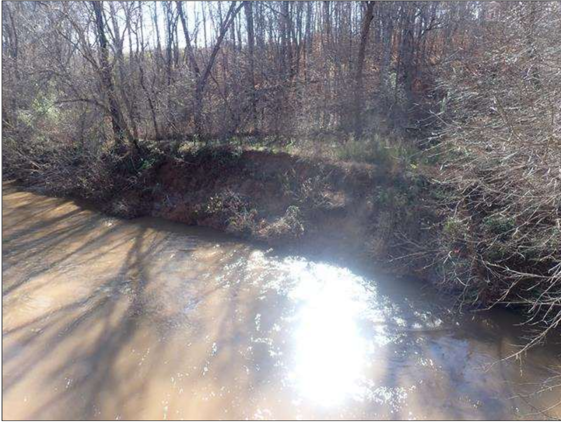
Channel and Channel Protection: southwest streambank 50ft from bridge, vertical cuts (70ft x 8ft x 12ft) with exposed tree roots
