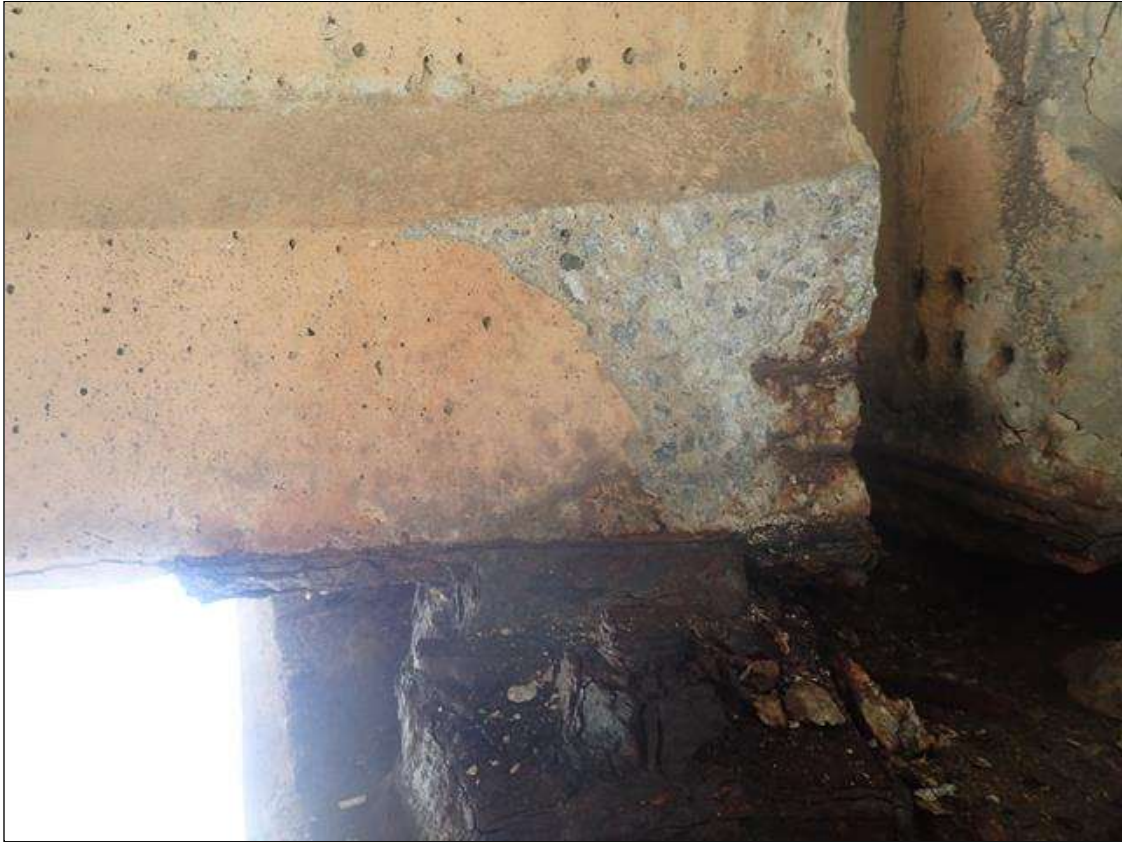
Span 3 Beam 3: (PAR) BOTTOM FLANGE LEFT SIDE AT BENT 2, SPALL (9IN X 8IN X 2-1/2IN) WITH EXPOSED RUSTED STRANDS
