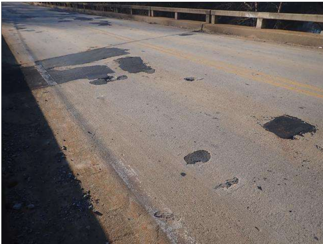
Span 4 Deck: BOTH LANES SCATTERED THROUGHOUT, PATCHED AREAS (UP TO 7FT X UP TO 12 FT)
