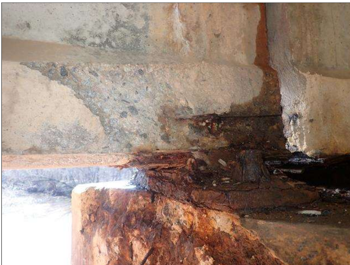
Span 4 Beam 4: (PAR) 24 INCHES X 8 INCHES X 2-1/2 INCHES DEEP SPALL WITH EXPOSED PRESTRESSING STRANDS ON LEFT SIDE OF BOTTOM FLANGE AT BENT 3
