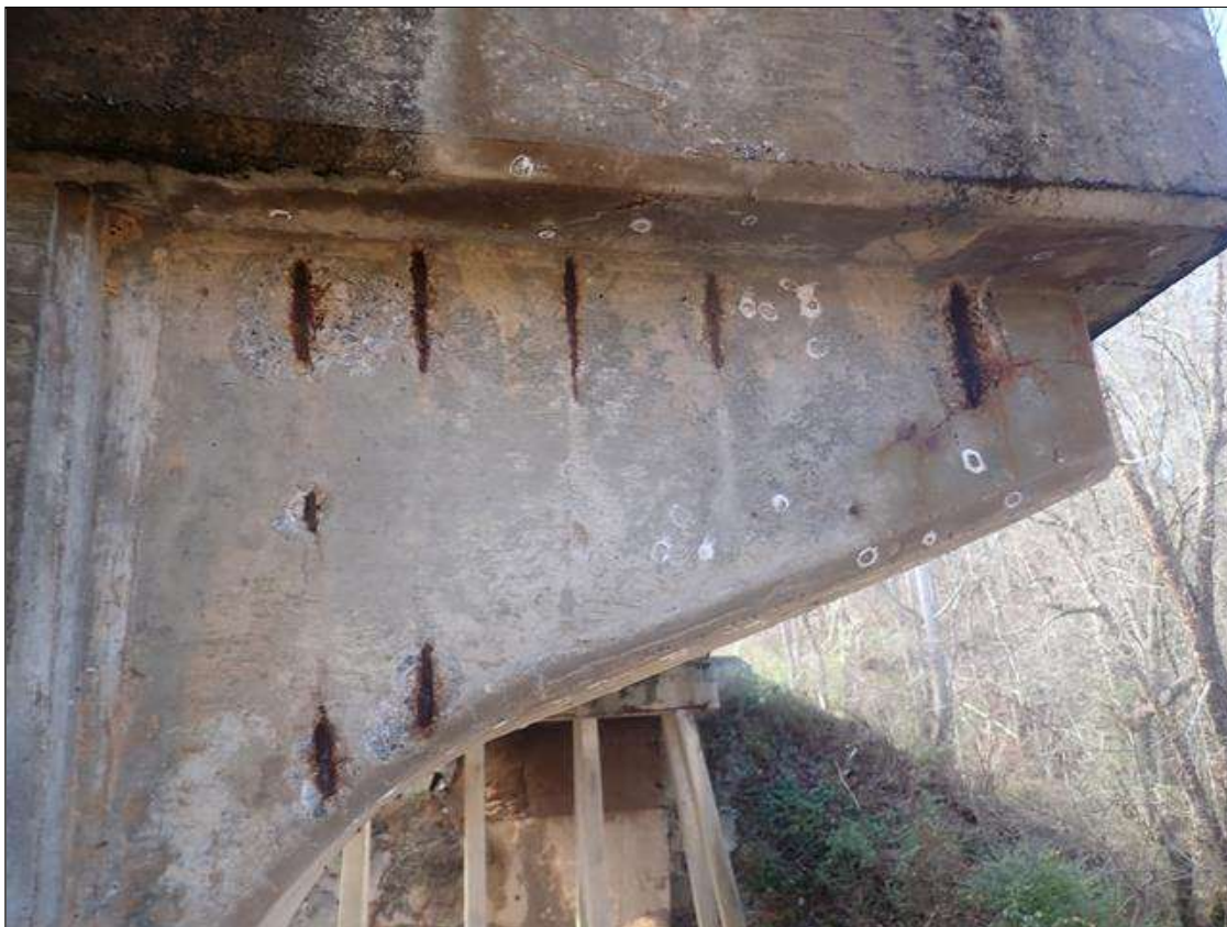
Bent 2 Cap 1: (8) UP TO 12 INCHES X 6 INCHES X 1/2 INCHES DEEP SPALLS WITH EXPOSED REBAR ON EAST FACE OF CORBEL AT NORTH END
