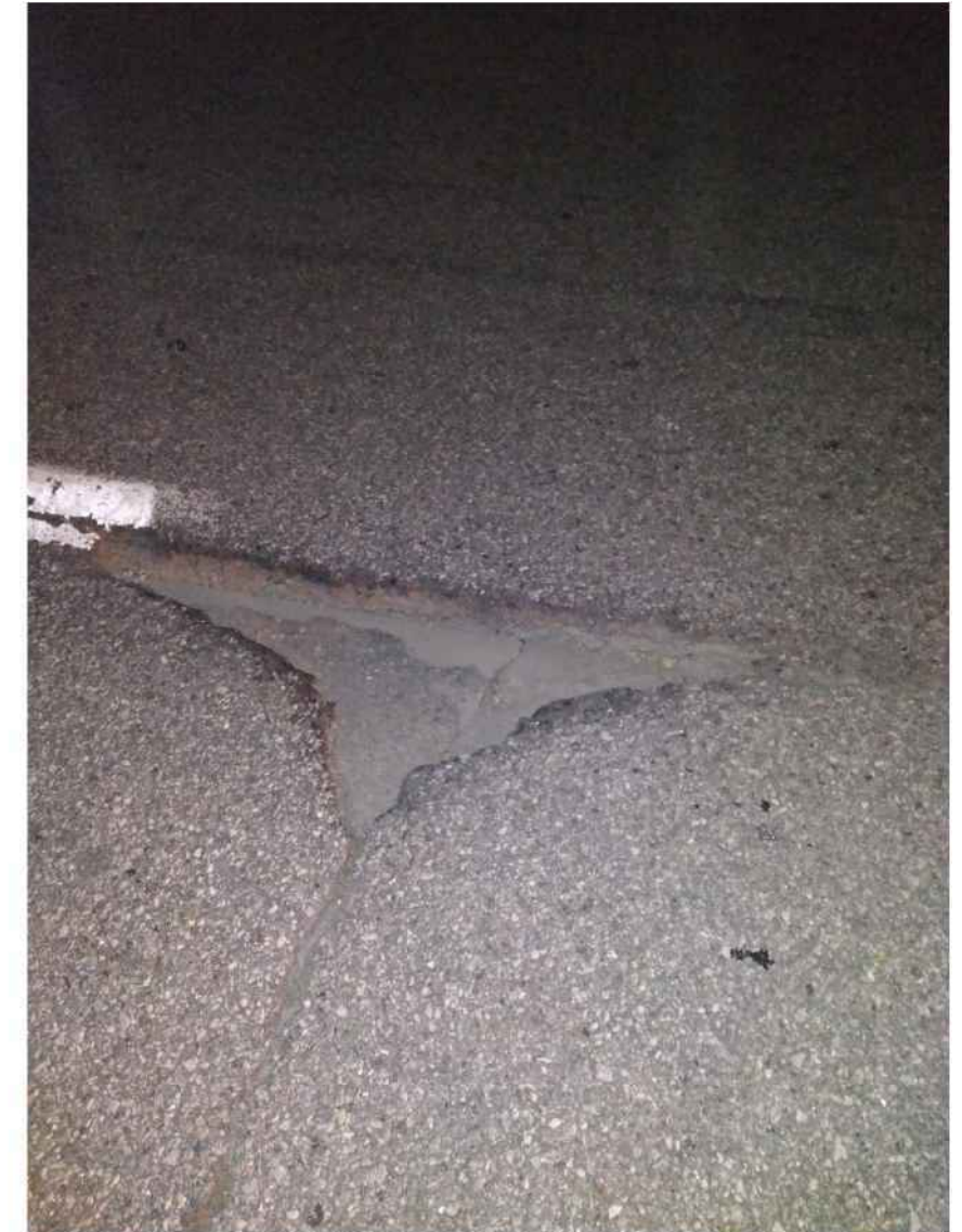
#13: REFLECTIVE CRACKING AT LONGITUDINAL AND TRANSVERSE JOINTS, SEVERE DEGRADATION OF OVERLAY, TYPICAL
