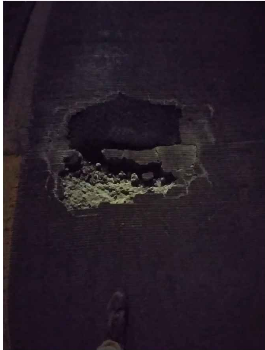
#8: SPALLING CONCRETE/POTHOLE AT TRANSVERSE JOINT, ATTEMPTED PATCH, TYPICAL
