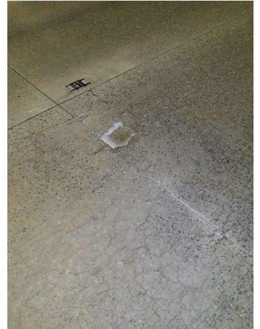
#7: CONCRETE DISTRESS – VERY FINE SPIDER WEB CRACKING AND TRANSVERSE JOINT SPALLING I-40 EB OSML
