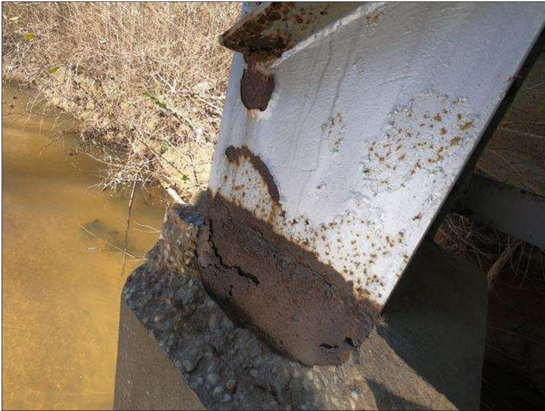
Bent 2 Pile 1: PAR: NEAR FLANGE PLATE AT CONCRETE ENCASEMENT ACTIVE CORROSION WITH SECTION LOSS 5" TALL X 12" WIDE, 7/16" REMAINING.
