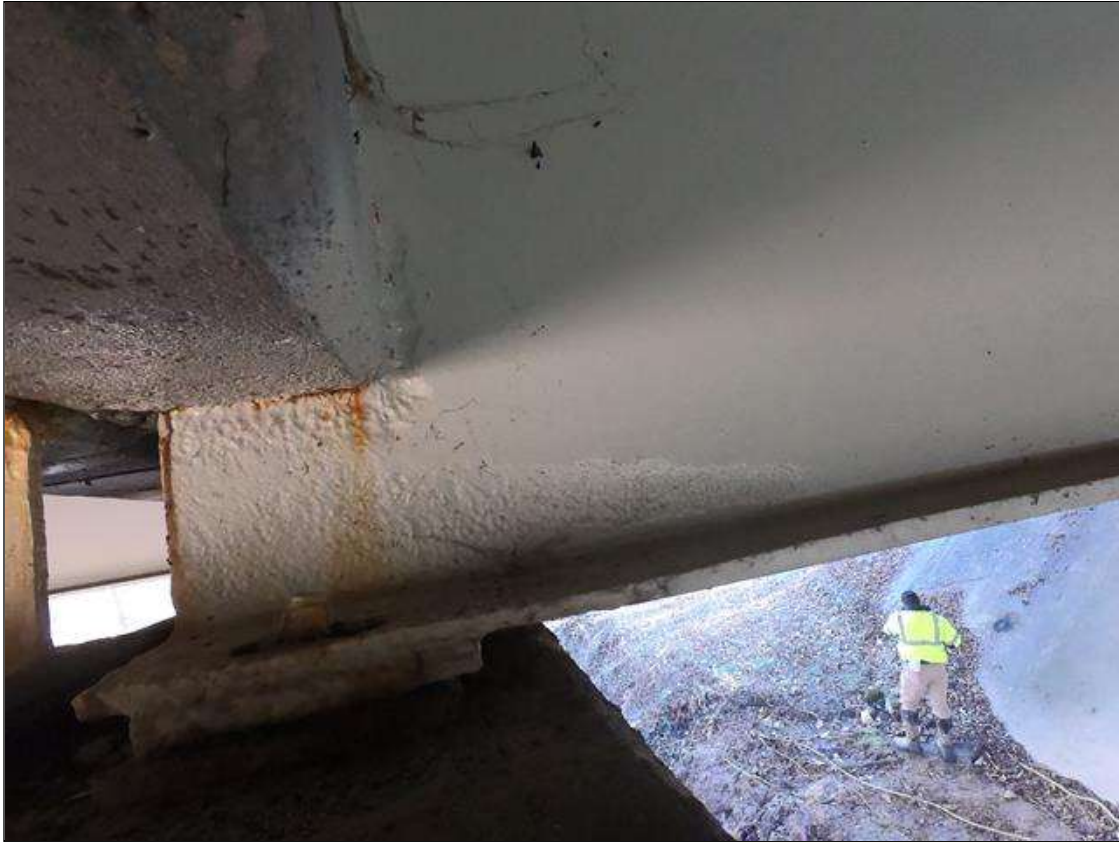
Span 1 Beam 2: PAR: ARRESTED CORROSION WITH SECTION LOSS AT BENT 1 IN WEB AROUND DIAPHRAGM, FOR 8" TALL X 2" WIDE WITH 7/16" OF WEB THICKNESS REMAINING, IN LOWER WEB FOR 3" TALL X 20" LONG WITH 7/16" OF WEB THICKNESS REMAINING, AND BOTTOM FLANGE FOR FULL WIDTH X 6" LONG WITH 1/2" OF FLANGE THICKNESS REMAINING
