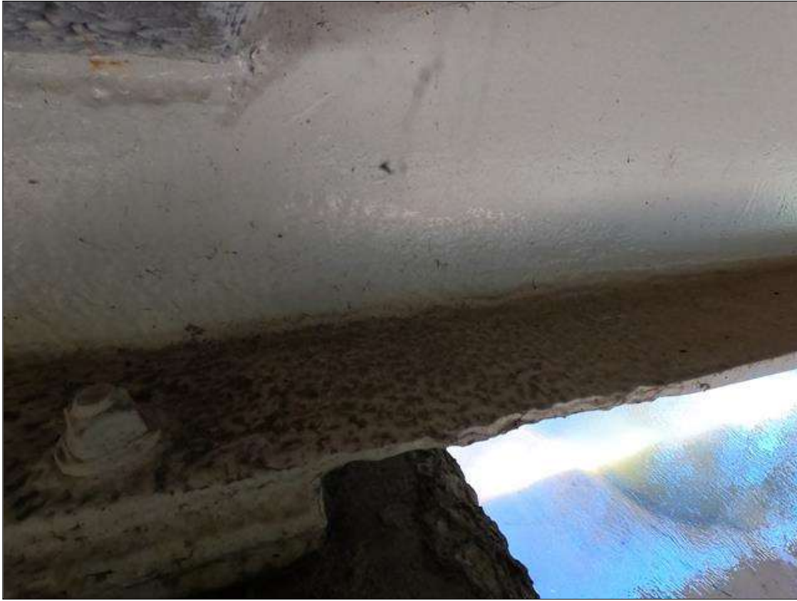
Span 2 Beam 3: PAR: ARRESTED CORROSION WITH SECTION LOSS AT BENT 2, IN LOWER WEB FOR 4" TALL X 34" LONG WITH 7/16" OF WEB THICKNESS REMAINING, IN BOTTOM FLANGE FOR FULL WIDTH X 12" LONG WITH 3/8" OF FLANGE THICKNESS REMAINING
