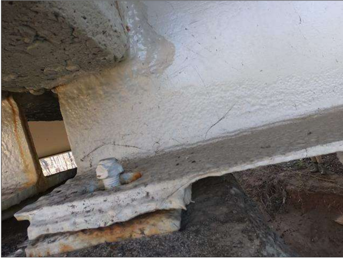
Span 1 Beam 1: PAR: AT BENT 1 SECTION LOSS WEB AROUND END DIAPHRAGM 1/4" REMAINING FOR 8" LONG X 2" TALL AND BOTH BOTTOM FLANGES 1/4" REMAINING, FULL WIDTH X 7" LONG
