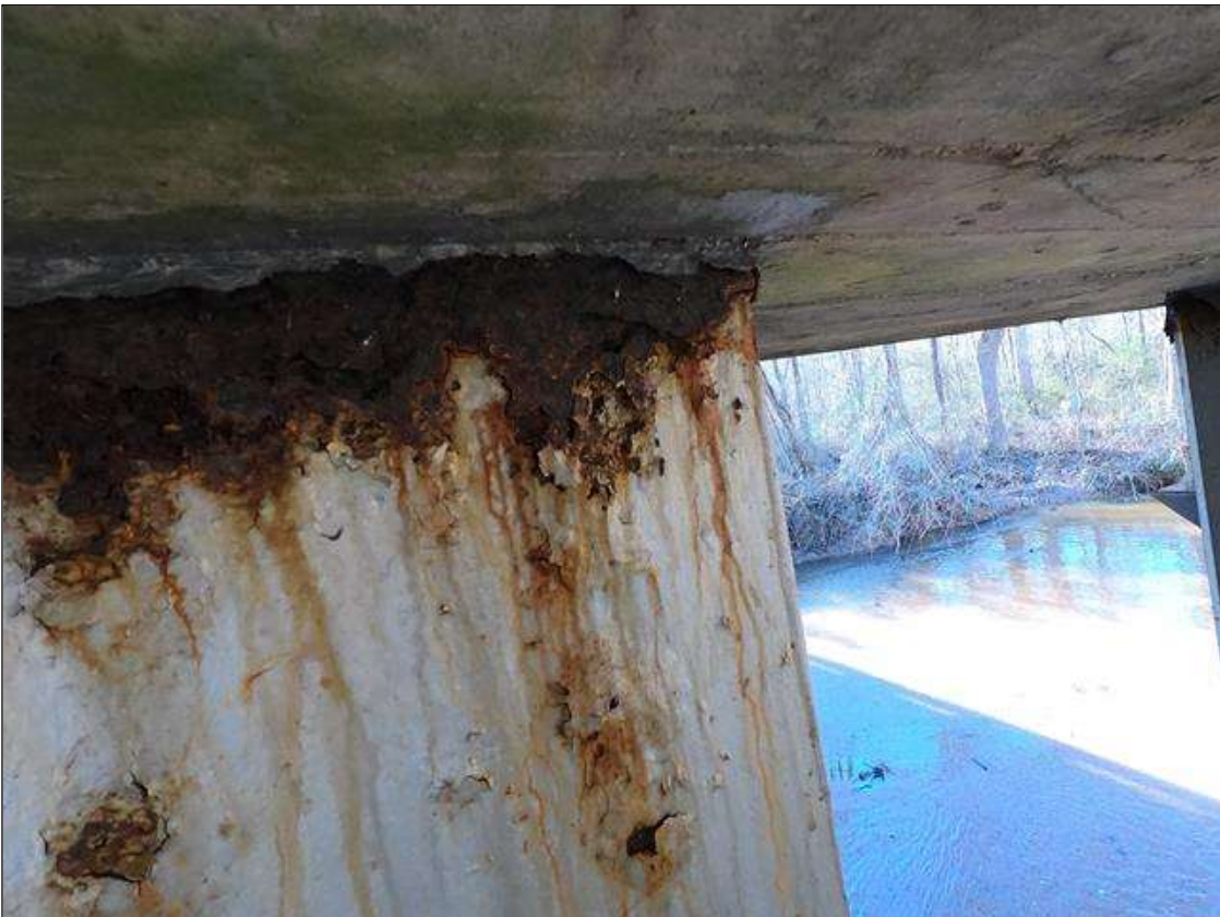
Bent 2 Pile 4: PAR: BENT 2 TOP OF PILE 4 ACTIVE CORROSION WITH SECTION LOSS 7/16" REMAINING X 12" WIDE X 2" TALL
