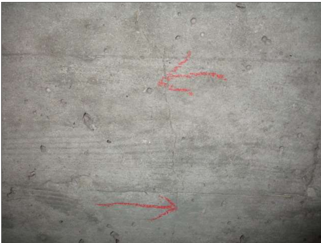
End Bent 1 Abutment: 1/32" VERTICAL CRACKING ALONG BACKWALL
