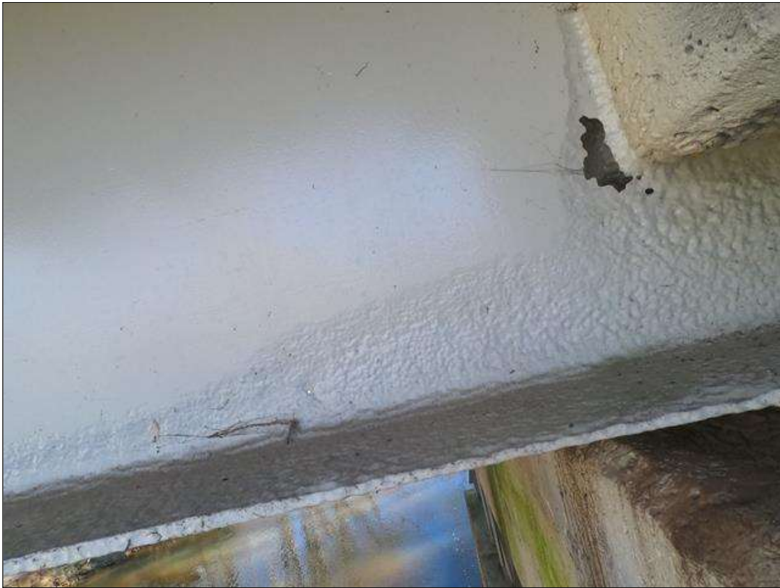
Span 2 Beam 1: PAR: 5" TALL X 2" WIDE AREA OF COMPLETE SECTION LOSS IN WEB AT END OF DIAPHRAGM AT BENT 1, 1/4" REMAINING ALONG BOTH BOTTOM FLANGES FOR 12" LONG X FULL WIDTH, AND 3/16" REMAINING ALONG LOWER 3" OF WEB FOR 12" LONG AT BENT 1
