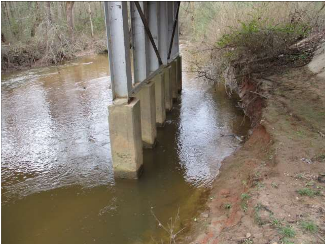
PAR: 15' LONG X 35' WIDE X 3' DEEP EROSION OF SPAN 3 SLOPE PROTECTION AROUND BENT 2 PILES
