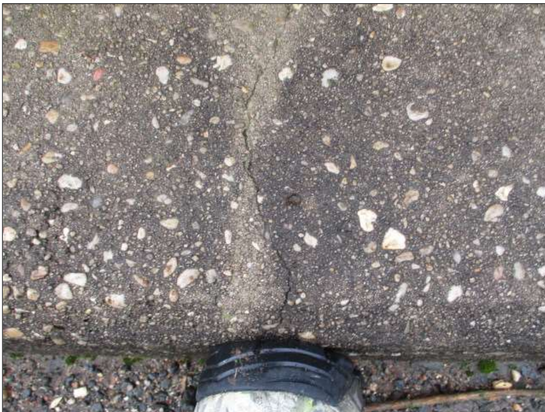
Span 3 Left Bridge Rail: 5 FULL WIDTH TRANSVERSE 1/32" CRACKS SCATTERED THROUGHOUT TOP OF PARAPET OF RAIL
