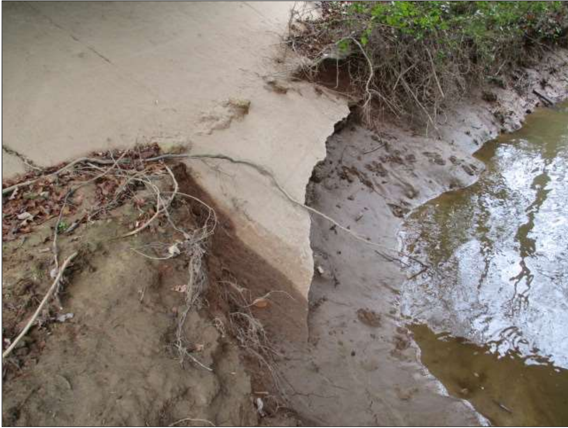
PAR: 13' WIDE X 8' LONG X 2' DEEP EROSION OF SPAN 1 SLOPE PROTECTION NEAR BENT 1
