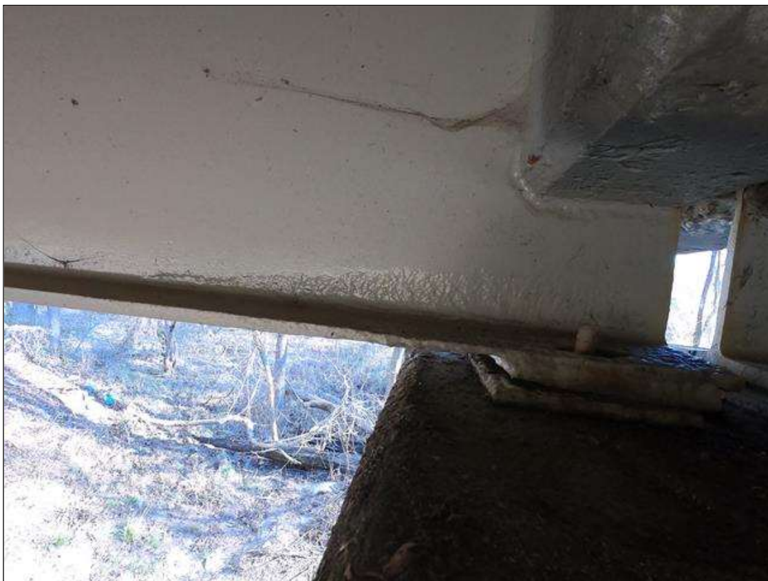
Span 3 Beam 4: PAR: AT BENT 2 SECTION LOSS LOWER WEB DOWN 7/16" REMAINING X 3" TALL X 36" LONG, AND BOTTOM FLANGE DOWN TO 3/8" REMAINING FULL WIDTH X 24" LONG, CORROSION ARRESTED.
