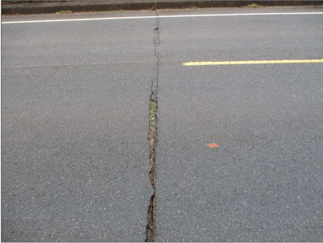
Span 2 Wearing Surface: FULL WIDTH TRANSVERSE CRACK UP TO 1/4" WIDE, WITH 1 SPALL UP TO 8 FT X 3" X 2" DEEP IN NORTH BOUND TRAVEL LANE AND 1 SPALL UP TO 9" X 4" X 2" DEEP IN SOUTH BOUND TRAVEL LANE, AT BENT 1
