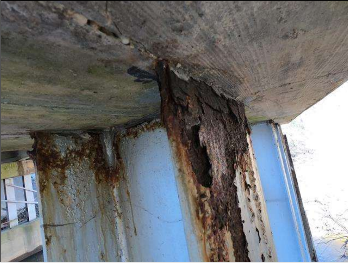
Bent 2 Pile 5: PAR: TOP OF PILE AT CAP ACTIVE CORROSION WITH SECTION LOSS 4" TALL X 12" WIDE X 1/4" REMAINING SECTION BOTH FLANGE PLATES AND WEB.
