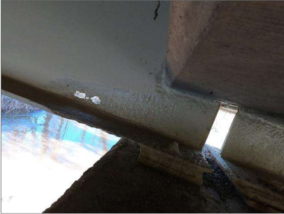
Span 2 Beam 1: PAR: 5" LONG X 2" TALL AREA OF 100% SECTION LOSS LOWER WEB, TWO RUSTED HOLES 1 FT FROM BENT 2, SECTION LOSS AREA UP TO 5" HIGH X 2.5 FT LONG IN BOTTOM OF WEB, CORROSION ARRESTED. AT BENT 2 IN BOTTOM FLANGE, 2 FT LONG X FULL WIDTH SECTION LOSS WITH 1/8" REMAINING, CORROSION ARRESTED.
