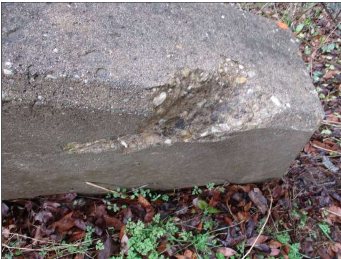
2' X 5" X 1" SPALL ON TOP OF SOUTHEAST WINGWALL
