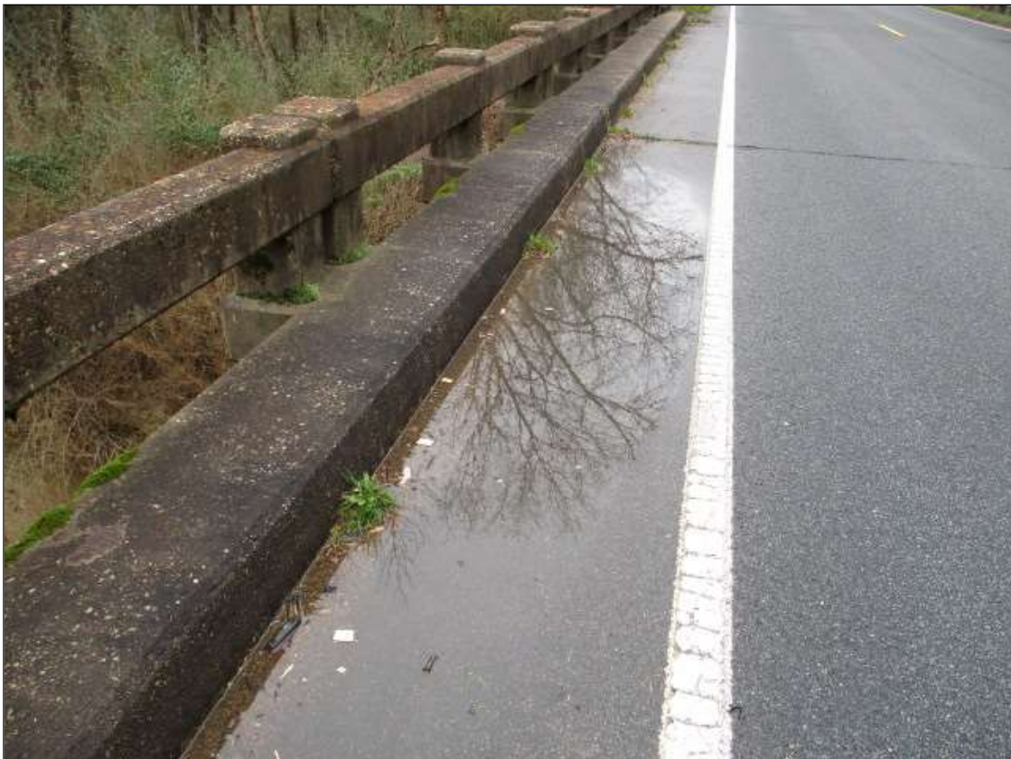
DEBRIS ALONG BOTH RAILS
