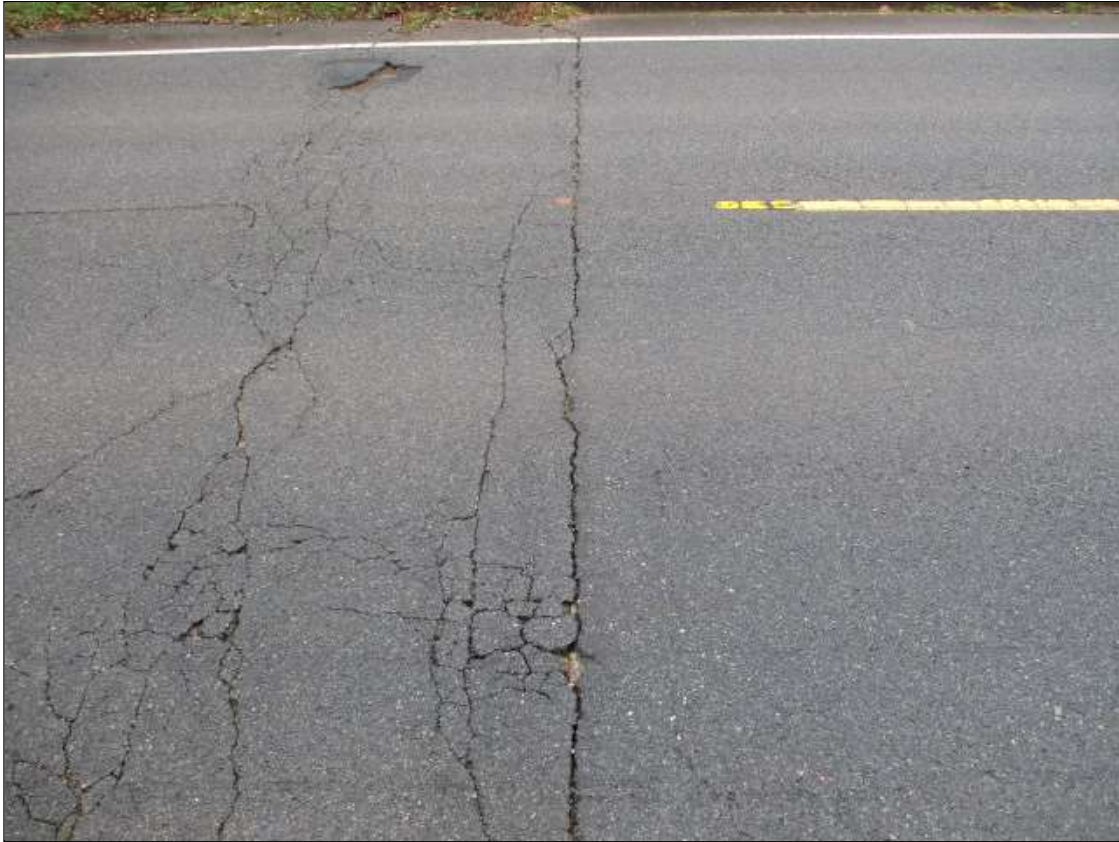
Span 1 Wearing Surface: FULL WIDTH TRANSVERSE CRACK UP TO 1/2" WIDE, WITH 3 SCATTERED SPALLS UP TO 1" DIAMETER X 1" DEEP SCATTERED ALONG THE LENGTH OF CRACK, AT END BENT 1
