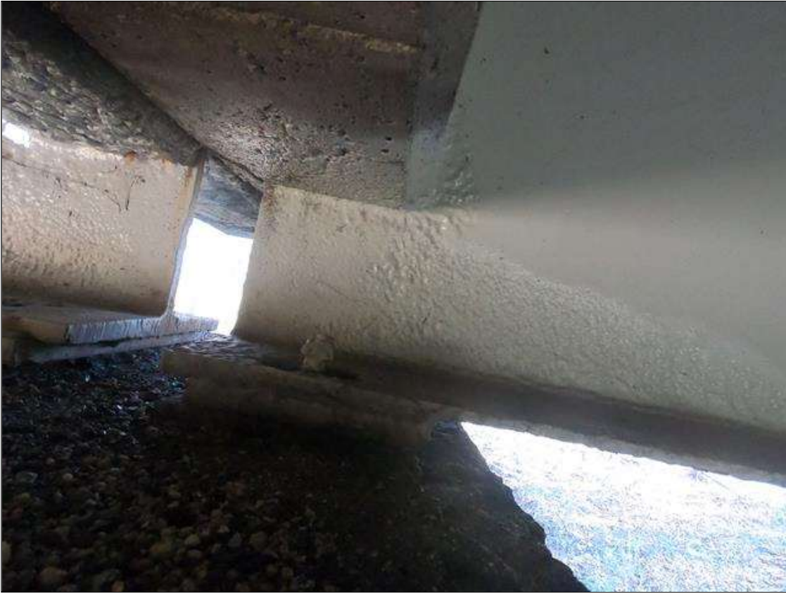
Span 1 Beam 4: PAR: AT BENT 1, SECTION LOSS IN WEB AROUND DIAPHRAGM 5/16" REMAINING 6" LONG X 2" WIDE, AND LOWER 3" X 24" LONG WITH 7/16" REMAINING, 3" X 24" LONG WITH 7/16" REMAINING, BOTTOM FLANGE SECTION LOSS DOWN TO 5/16" REMAINING X 16" LONG X FULL WIDTH, CORROSION ARRESTED.
