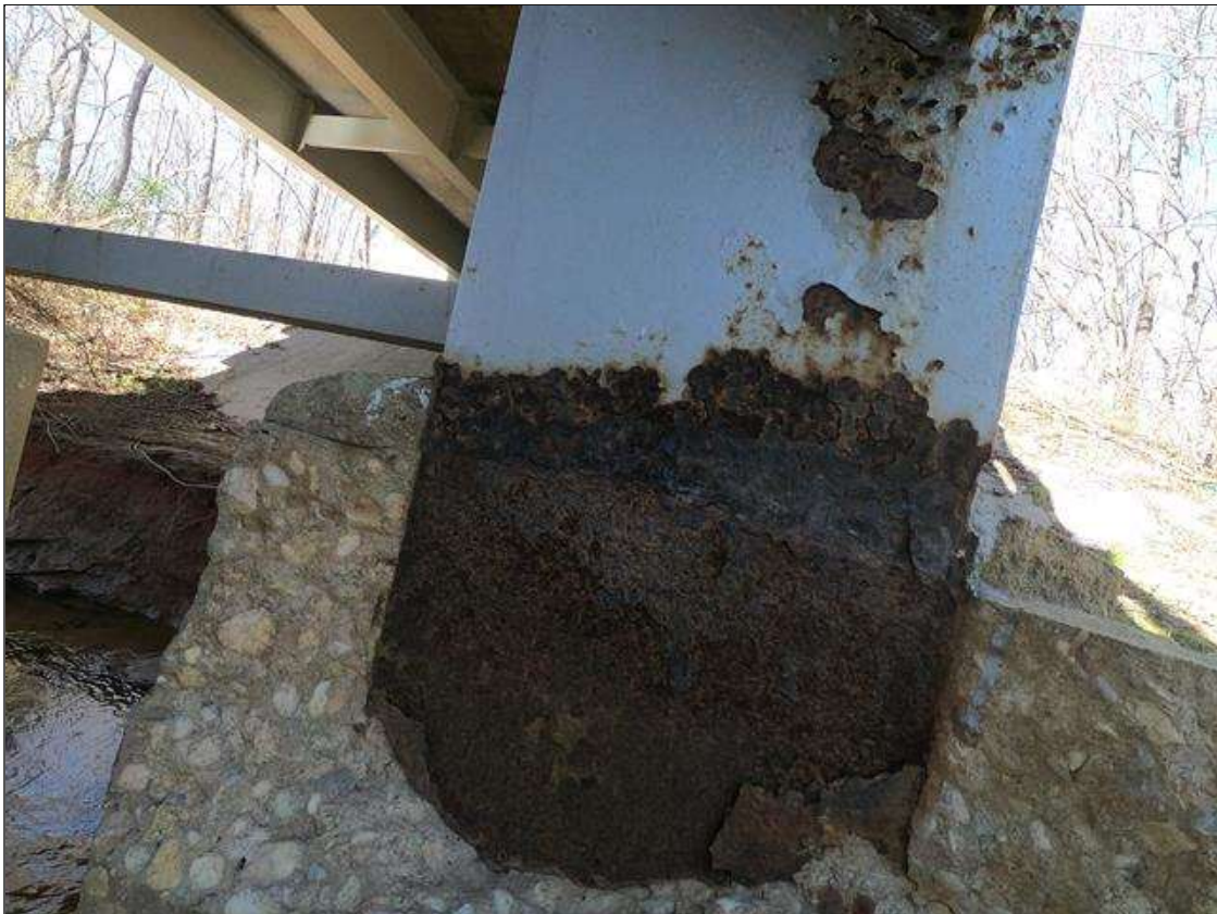
Bent 2 Pile 6: PAR: NEAR FLANGE PLATE AT CONCRETE ENCASEMENT: ACTIVE CORROSION WITH SECTION LOSS 1/4" REMAINING 12" WIDE X 8" TALL
