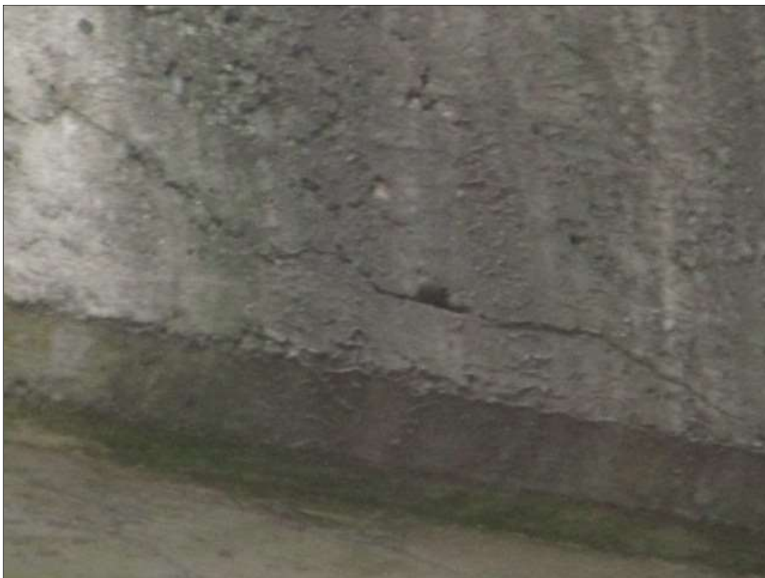
Bent 1 Cap 1: 3 FT LONG LONGITUDINAL CRACK UP TO 1/16" WIDE IN TOP OF NORTH FACE OF CAP ABOVE PILE 1 AND 6
