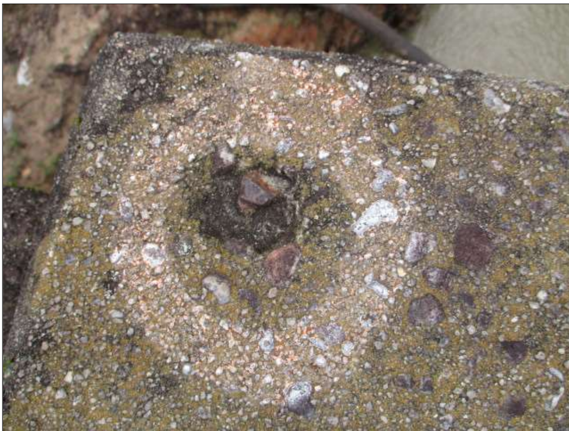
Span 2 Right Bridge Rail: 1" DIAMETER X 3/4" DEEP SPALL WITH EXPOSED REBAR ON TOP OF POST 8
