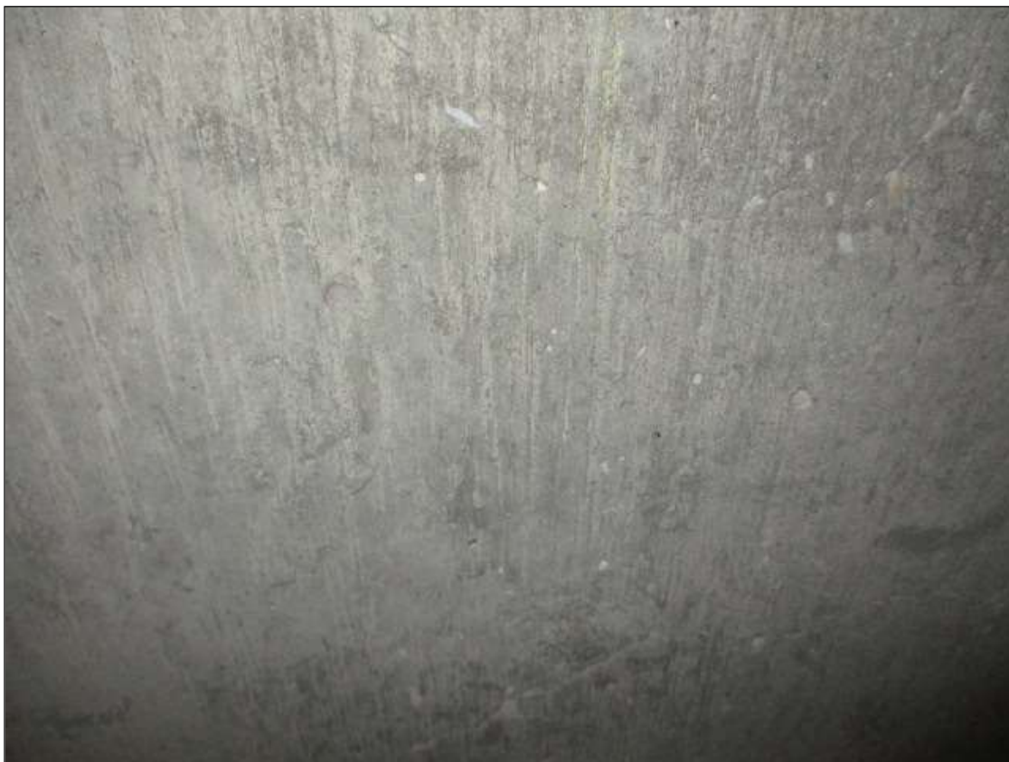
Span 1 Deck: 1/64" MAP CRACKING WITH EFFLORESCENCE SCATTERED THROUGHOUT UNDERSIDE OF DECK IN ALL BAYS
