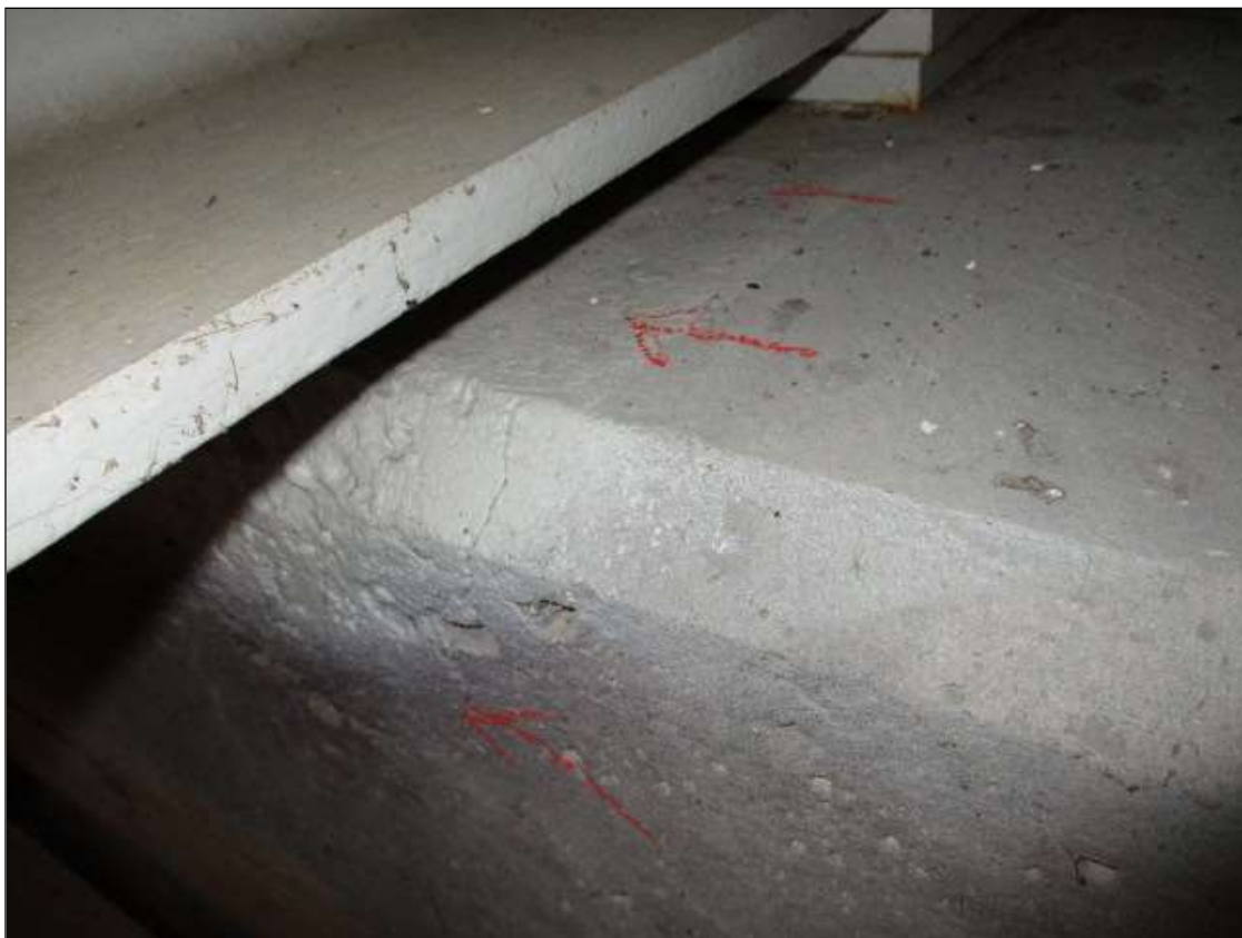
End Bent 1 Cap 1: 1/32" VERTICAL AND HORIZONTAL CRACKING
