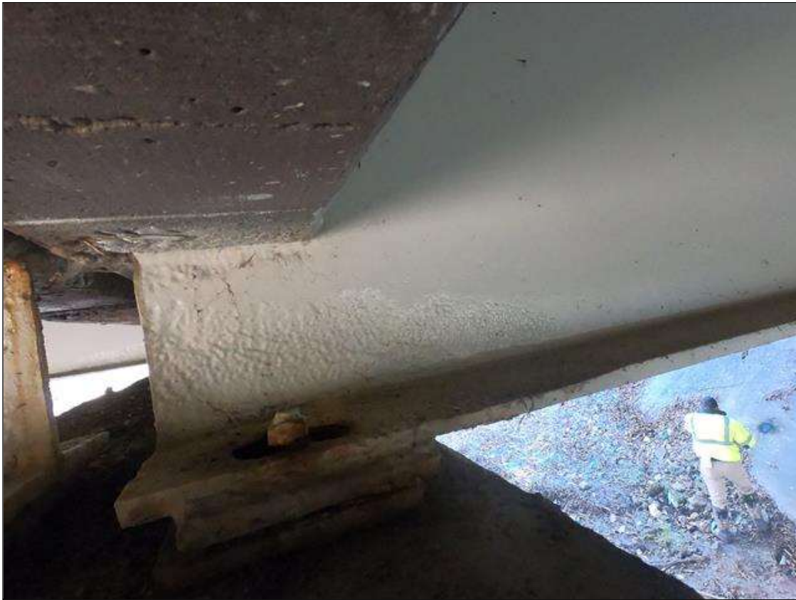
Span 1 Beam 3: PAR: AT BENT 1, SECTION LOSS IN WEB AROUND DIAPHRAGM 3/8" REMAINING 8" LONG X 1" WIDE, LOWER 5" X 20" LONG WITH 7/16" REMAINING, BOTTOM FLANGE SECTION LOSS DOWN TO 1/2" REMAINING X 8" LONG X FULL WIDTH, CORROSION ARRESTED
