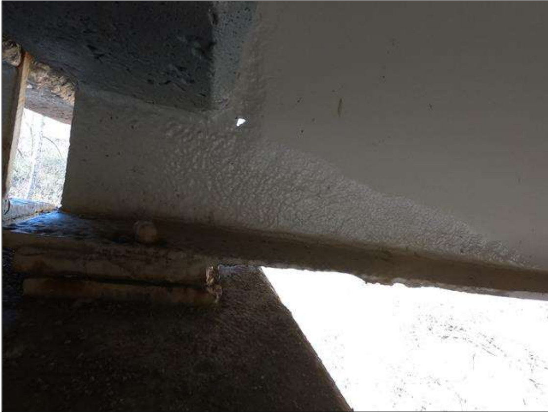
Span 3 Beam 1: PAR: AT BENT 2, SECTION LOSS 7/16" REMAINING LOWER WEB 6" X 30" LONG, AROUND END DIAPHRAGM IN WEB 7" LONG X 1" WIDE WITH 1/2" DIAMETER RUST HOLE, AND BOTTOM FLANGE DOWN TO 1/4" REMAINING FULL WIDTH X 16" LONG, CORROSION ARRESTED
