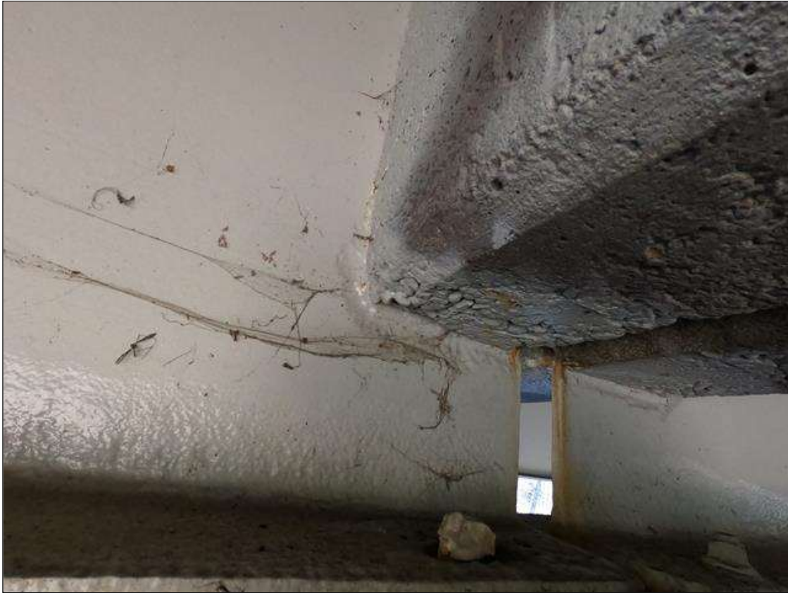
Span 3 Beam 3: PAR: ARRESTED CORROSION WITH SECTION LOSS IN BEAM AT BENT 2, IN BOTTOM FLANGE FOR FULL WIDTH X 24" LONG WITH 7/16" OF FLANGE THICKNESS REMAINING, AND IN WEB AROUND DIAPHRAGM FOR 8" LONG X 1" WIDE X 7/16" REMAINING
