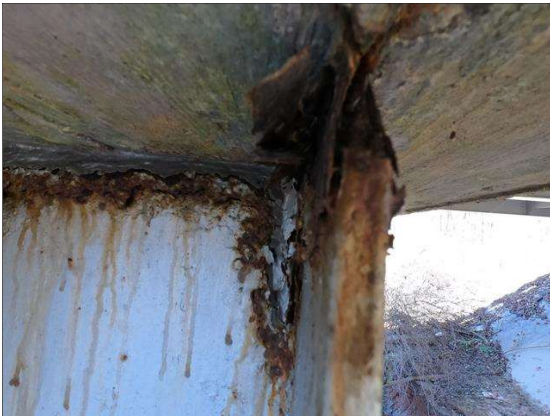
Bent 2 Pile 6: PAR: TOP OF PILE AT CAP: FAR FLANGE PLATE ACTIVE CORROSION WITH SECTION LOSS 6" WIDE X 1" TALL, DOWN TO 1/4" REMAINING.
