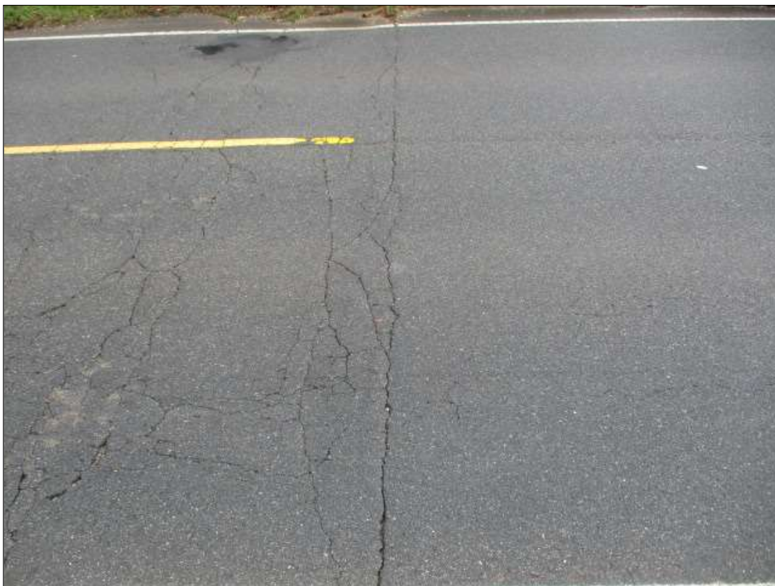
Span 3 Wearing Surface: FULL WIDTH TRANSVERSE CRACK UP TO 1/2" WIDE, WITH SCATTERED SPALLS UP TO 1" DIAMETER X 1" DEEP SCATTERED ALONG THE LENGTH OF CRACK, AT END BENT 2
