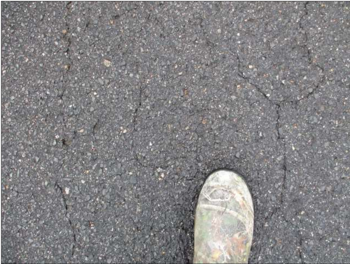
Span 1 Wearing Surface: 1/16" MAP CRACKING IN TRAVEL LANES
