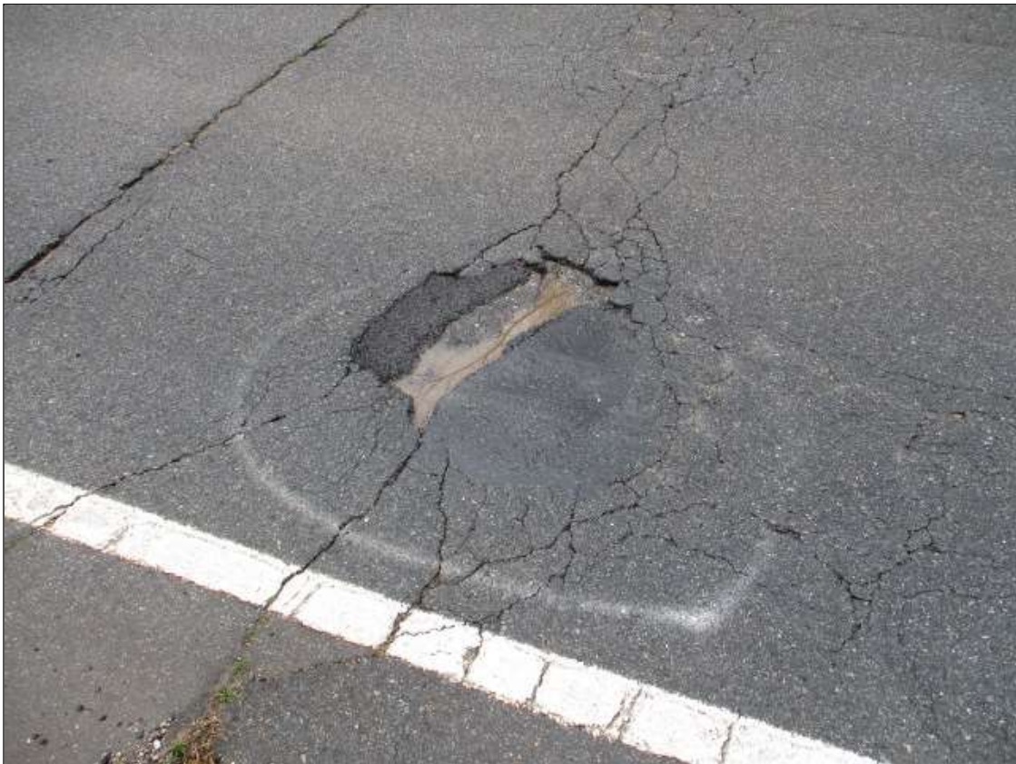
3' X 1' X 2 1/2" DEEP POTHOLE IN SOUTH APPROACH AT SOUTH BOUND LANE
