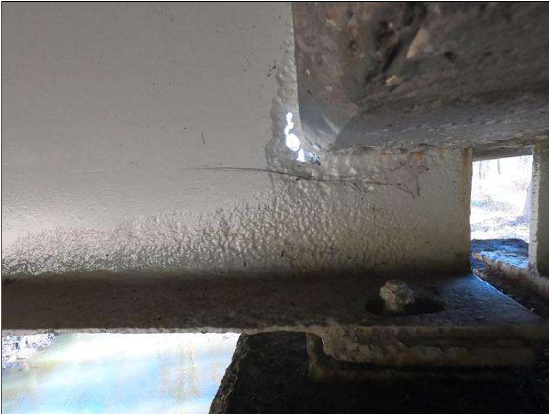
Span 2 Beam 4: PAR: AT BENT 1, SECTION LOSS IN WEB AROUND DIAPHRAGM 5/16" REMAINING FOR 8" LONG X 2.5" WIDE WITH RUST HOLE 3" X 1" LOCATED AT 6" FROM BEARING, LOWER 3" X 24" LONG WITH 7/16" REMAINING IN WEB, AND SECTION LOSS IN BOTTOM FLANGE DOWN TO 3/16" REMAINING FOR 36" LONG X FULL WIDTH, CORROSION ARRESTED
