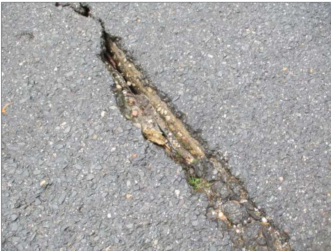
Span 3 Wearing Surface: 16" X 4" X 2" DEEP POTHOLE IN NORTH BOUND LANE OVER BENT 2
