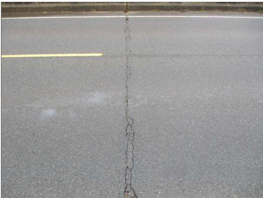
Span 3 Wearing Surface: FULL WIDTH TRANSVERSE CRACK UP TO 1/4" WIDE OVER BENT 2
