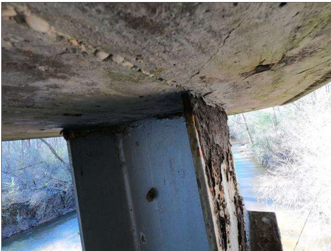
Bent 2 Pile 1: PAR: TOP OF PILE FAR FLANGE PLATE ACTIVE CORROSION WITH SECTION LOSS 1/4" REMAINING 2" TALL X 12" WIDE
