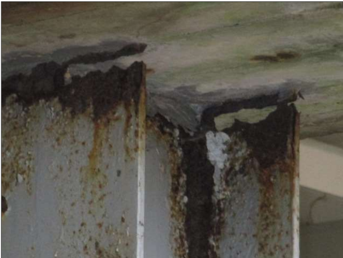
Bent 1 Pile 9: PAR: TOP OF PILE ACTIVE CORROSION BOTH DOWNSTREAM FLANGE PLATES WITH COMPLETE SECTION LOSS 5-1/2" X 1", AND SECTION LOSS WITH 3/8" REMAINING 6-1/2" X 2".
