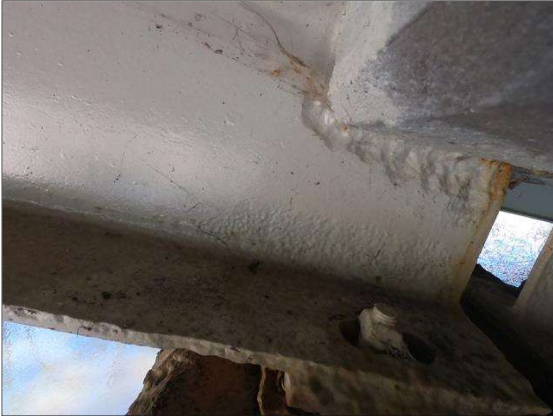
Span 2 Beam 3: PAR: AT BENT 1, SECTION LOSS IN WEB AROUND DIAPHRAGM 3/8" REMAINING 8" LONG X 2" WIDE, AND LOWER 5" X 13" LONG WITH 7/16" REMAINING, BOTTOM FLANGE SECTION LOSS DOWN TO 1/2" REMAINING X 8" LONG X FULL WIDTH, CORROSION ARRESTED.
