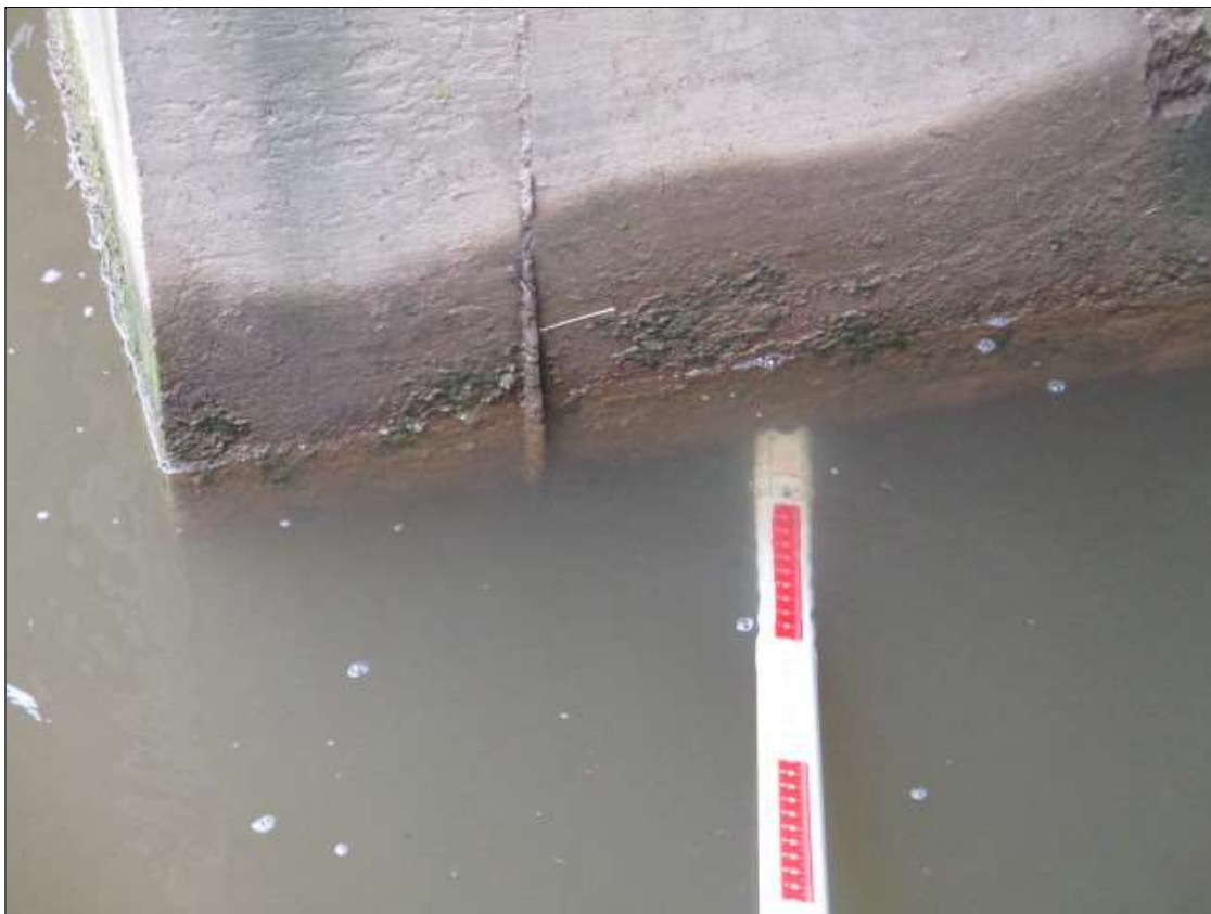
BENT 1 CONCRETE PILE ENCASEMENT IS NOT TOUCHING THE STREAMBED
