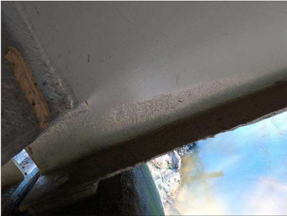
Span 2 Beam 4: PAR: AT BENT 2 SECTION LOSS BOTTOM FLANGE DOWN TO 5/16" REMAINING FULL WIDTH X 24" LONG, AND LOWER WEB DOWN TO 3/8" REMAINING FOR 6" TALL X 36" LONG, CORROSION ARRESTED
