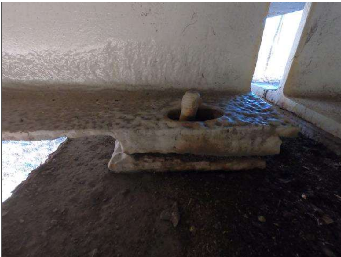
Span 3 Beam 4 - Near Bearing: PAR: COMPLETE SECTION LOSS IN LEFT ANCHOR BOLT NUT
