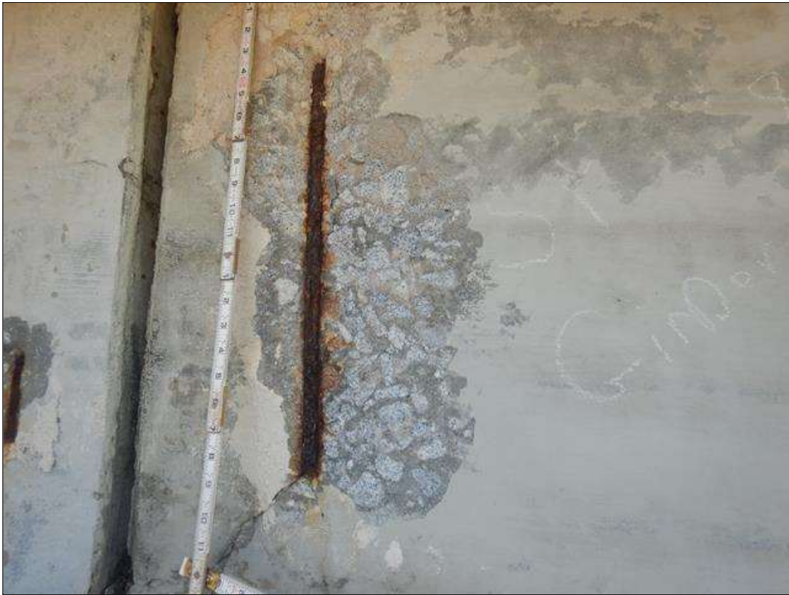
Span 8 Beam 1: 22" HIGH X UP TO 10" WIDE X 1" DEEP SPALL WITH EXPOSED REINFORCEMENT WITH NO MEASURABLE SECTION LOSS IN FORMERLY PATCHED AREA IN NORTH FACE, AT BENT 8
