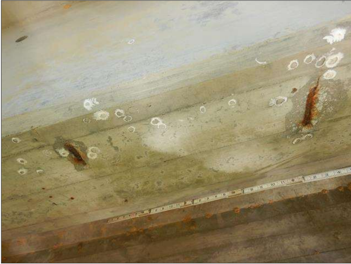
Span 8 Beam 4: (2) SPALLS ON UNDERSIDE OF BEAM LOCATED 12' AND 14' FROM BENT 8. 5" LONG X 6" WIDE X 1/2" DEEP AND 3" LONG X 4" WIDE X 1/2" DEEP, BOTH WITH EXPOSED REINFORCEMENT. NO MEASURABLE SECTION LOSS
