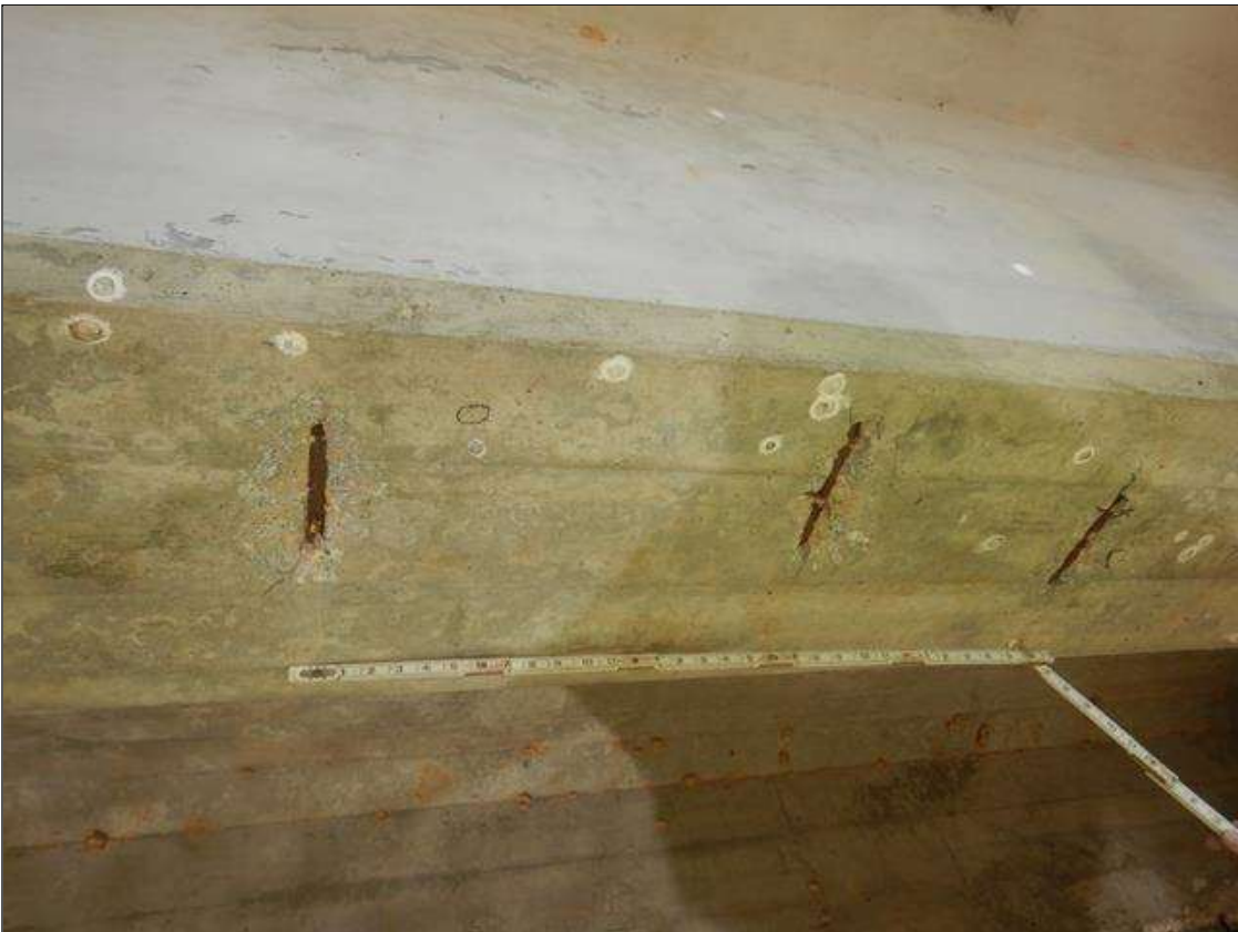
Span 3 Beam 4: THREE (3) 8" LONG X 3" WIDE X 1/2" DEEP SPALLS WITH EXPOSED REINFORCEMENT WITH NO MEASURABLE LOSS IN UNDERSIDE OF BEAM, STARTING AT 8 FT FROM BENT 3.
