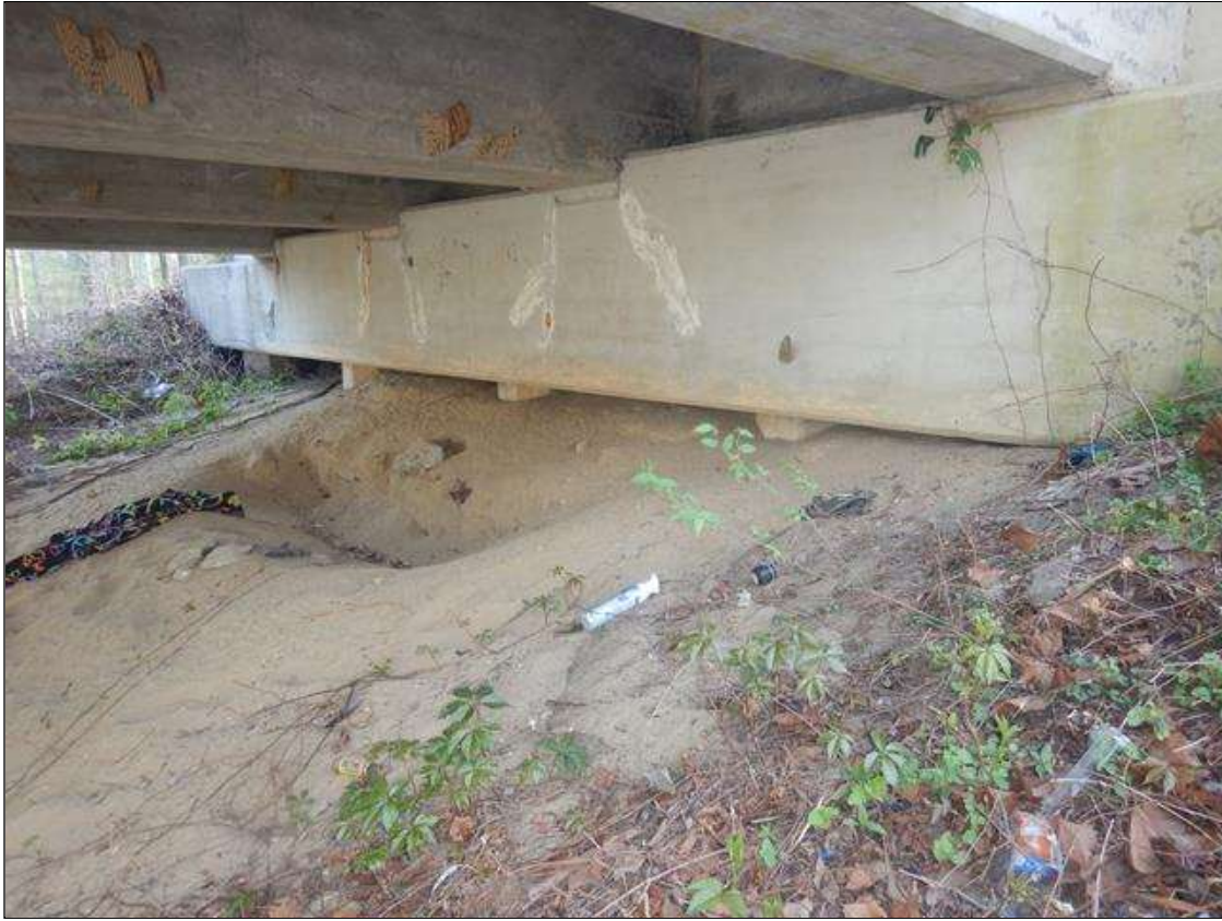
End bent 1 Abutment: PAR: 25' LONG X UP TO 15" HIGH X UP TO FULL DEPTH VOID UNDER CAP WITH PILES 2-5 EXPOSED
