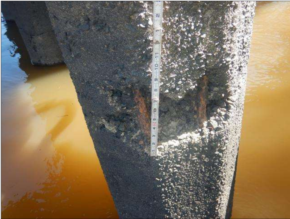
Bent 8 Pile 5: PAR: 18" WIDE X 10" HIGH X 3" DEEP SPALL WITH EXPOSED REBAR WITH NO MEASURABLE SECTION LOSS ON SOUTH FACE, 3' ABOVE WATERLINE
