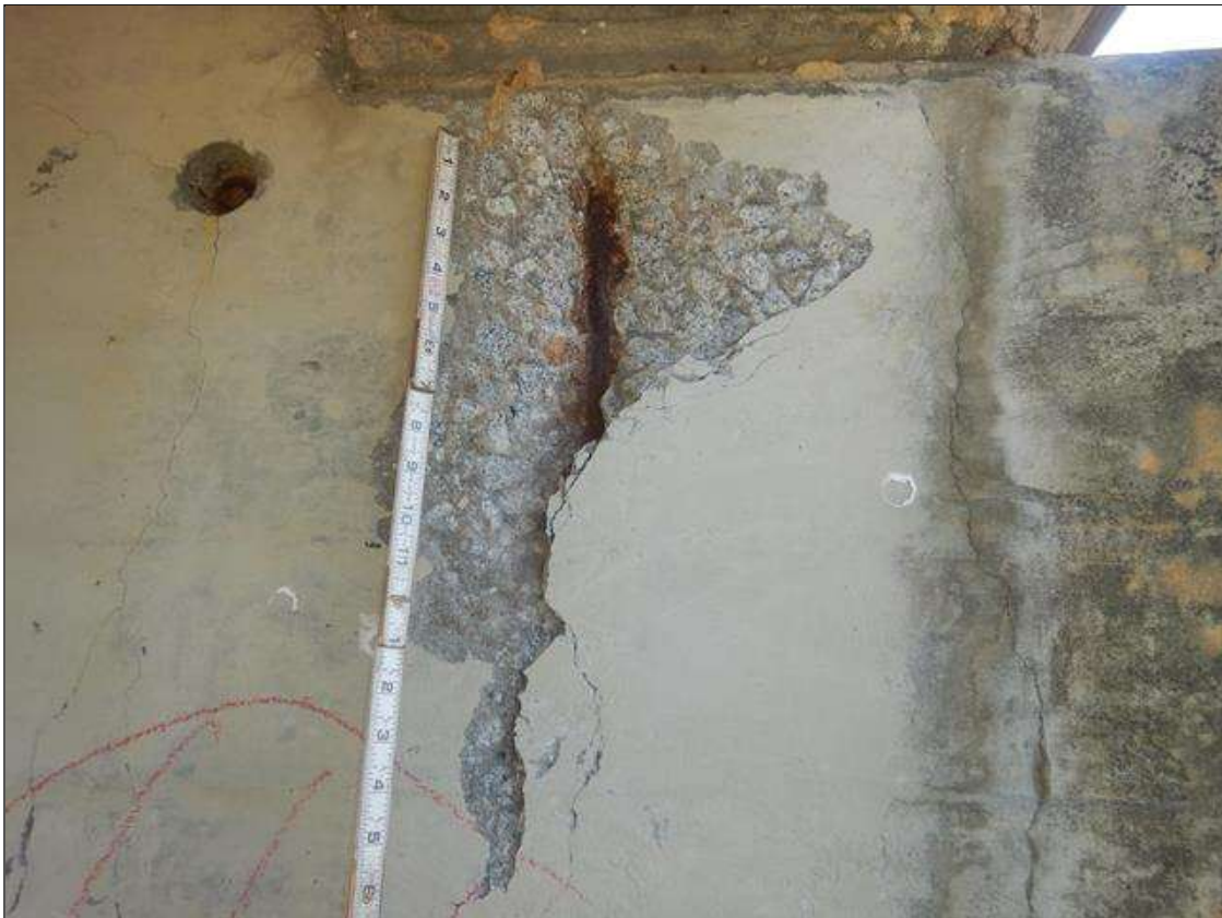
Bent 8 Cap 1: PAR: 1'-7" HIGH X 1' WIDE X 1 1/4" DEEP SPALL WITH EXPOSED REINFORCING ON WEST FACE BELOW BEAM 4, NO MEASURABLE SECTION LOSS
