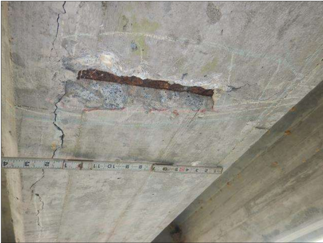
Span 10 Beam 3: PAR: 5' LONG X 18" WIDE AREA OF SPALLS WITH EXPOSED REINFORCEMENT AND UP TO 1/16" WIDE LONGITUDINAL CRACKS, STARTING 6' FROM END BENT 2 ON UNDERSIDE OF BEAM. SPALL SIZES VARY FROM 3" LONG X 6" WIDE X 1" DEEP TO 1'-6" LONG X 1' WIDE X 1 1/4" DEEP
