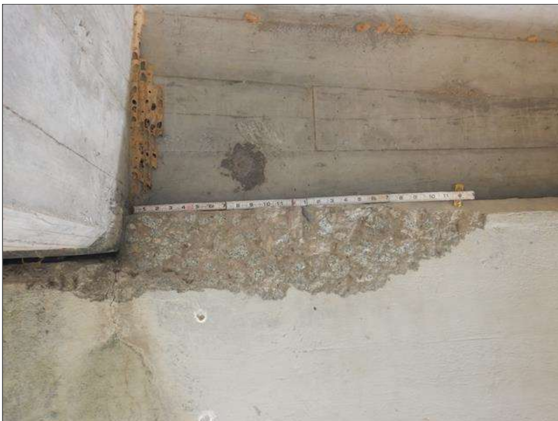
Bent 4 Cap 1: 2'-5" LONG X 6" HIGH X UP TO 4" DEEP SPALL IN TOP OF CAP, WEST FACE, BAY 1.
