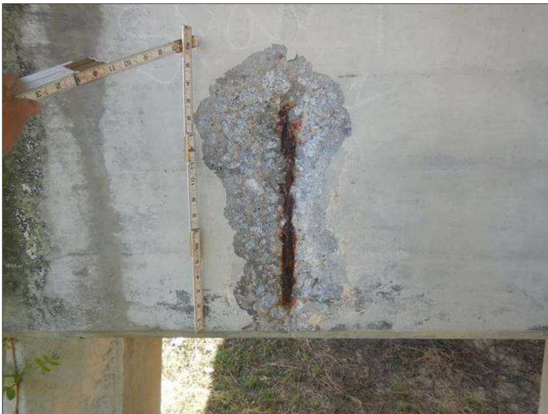
Bent 9 Cap 1: 1'-7" HIGH X 9 1/2" WIDE X 2" DEEP SPALL WITH EXPOSED REINFORCEMENT ON WEST FACE BELOW BEAM 1, NO MEASURABLE SECTION LOSS
