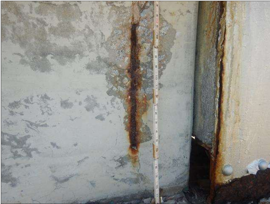
Span 7 Beam 1: 8" LONG X 1'-9" HIGH X UP TO 1" DEEP SPALL WITH EXPOSED REINFORCEMENT NO MEASURABLE SECTION LOSS IN NORTH FACE, AT BENT 6.
