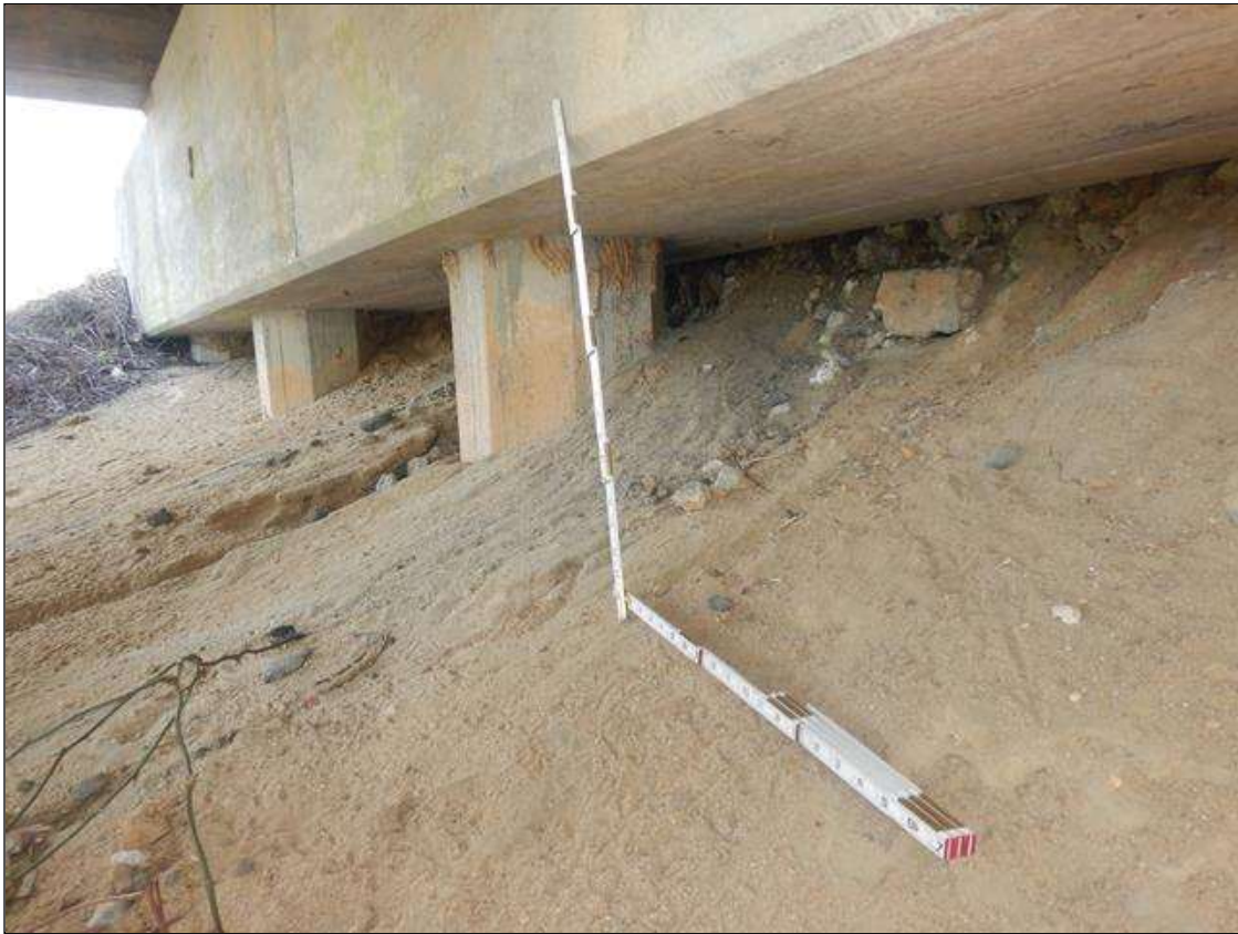
End bent 2 Abutment: PAR: FULL LENGTH X UP TO 1'-8" HIGH X FULL DEPTH VOID UNDER CAP WITH ALL PILES EXPOSED. THERE IS A TIMBER BACKWALL IN PLACE BEHIND PILES 4-5. THERE IS NO RETAINING MEASURE IN PLACE TO HOLD BACK FILL FOR THE REMAINDER OF CAP LENGTH
