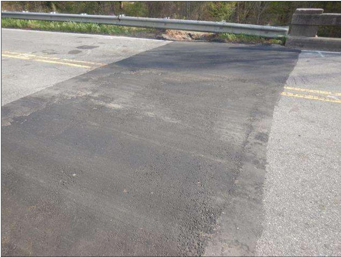
12' LONG X FULL WIDTH WEDGE PATCH HAS BEEN ADDED TO THE EAST APPROACH ROADWAY SINCE PREVIOUS INSPECTION
