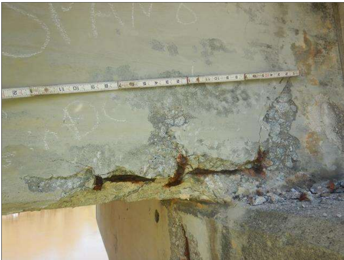
Span 8 Beam 4: PAR: 2' LONG X 1' HIGH X 6 1/2" WIDE ON BOTTOM FACE X 1 1/2" DEEP SPALL WITH EXPOSED REBAR, LOCATED ON BOTTOM RIGHT CORNER OVER BENT 8
