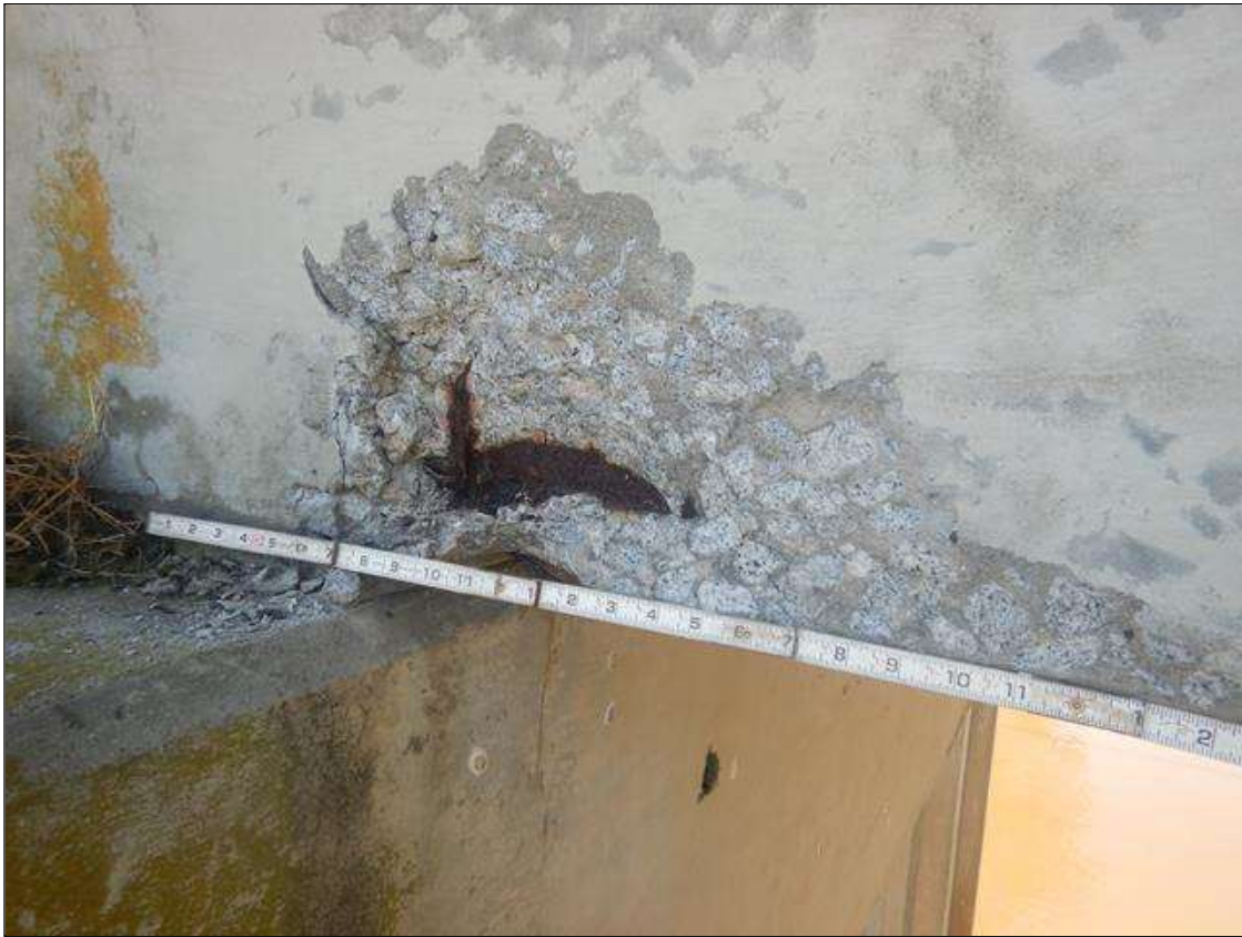
Span 7 Beam 1: 1'-3" LONG X 11" HIGH X 3/4 IN DEEP SPALL WITH EXPOSED REINFORCEMENT NO MEASURABLE SECTION LOSS, LOCATED IN NORTH FACE ABOVE BENT 7 CAP.
