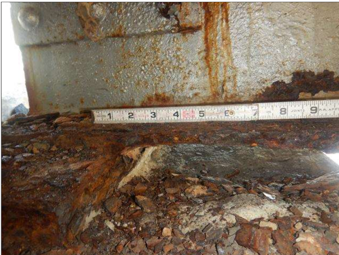
Span 6 Beam 5: PAR: 7" LONG X 2" WIDE AREA OF CORROSION WITH 3/8" SECTION LOSS ON NORTH SIDE OF BOTTOM FLANGE AT BENT 6. 5/8" REMAINING
