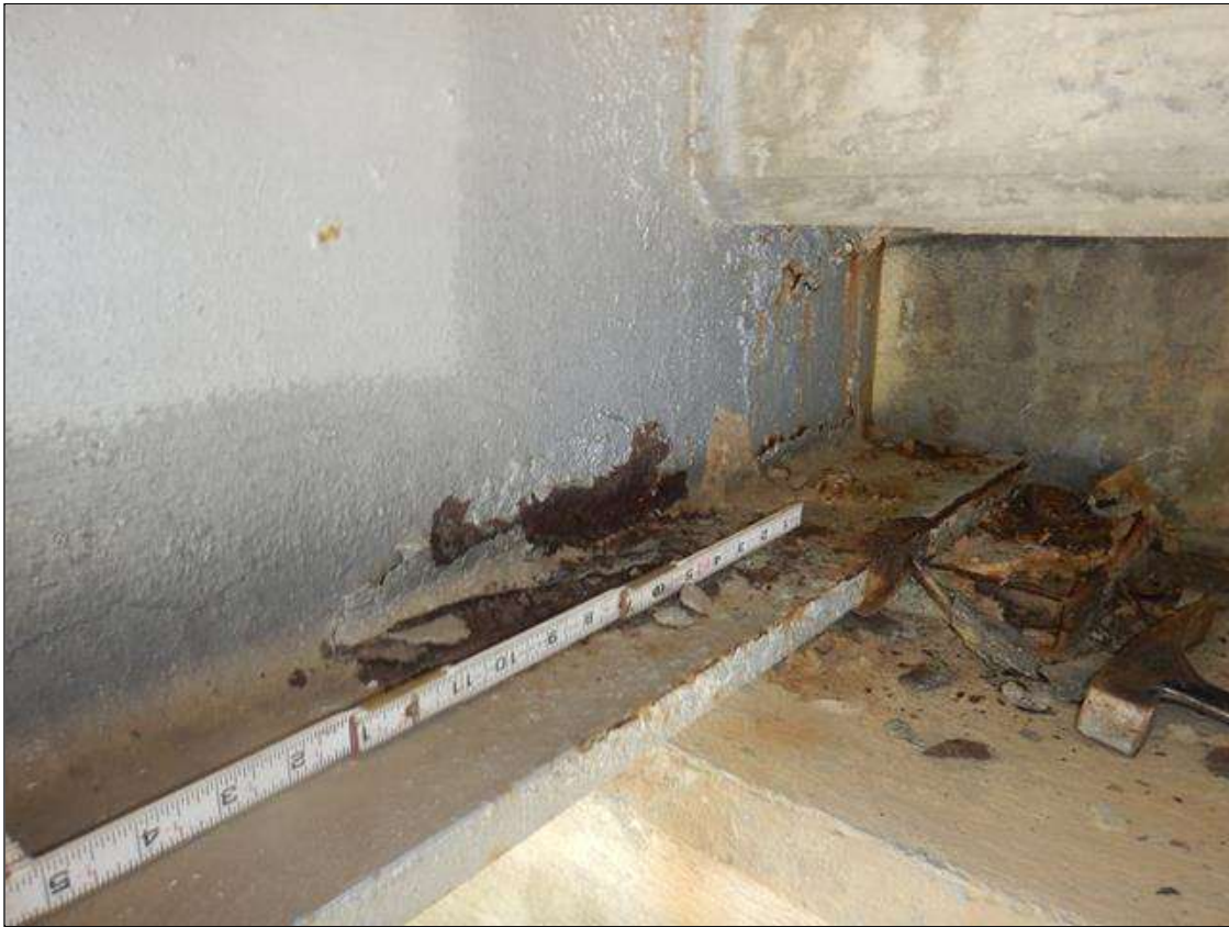
Span 6 Beam 2: 6" LONG X FULL WIDTH AREA OF SURFACE CORROSION WITH MINOR DELAMINATION ON BOTTOM FLANGE AND BOTTOM 3 IN OF WEB IN SOUTH FACE AT BENT 6 BEAM END. NO MEASURABLE SECTION LOSS NOTED.
