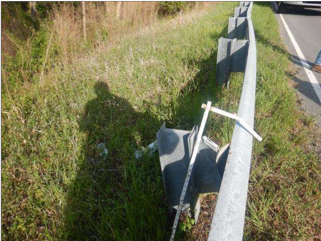
PAR: MODERATE AREA OF IMPACT DAMAGE ON NORTHWEST GUARDRAIL STARTING APPROXIMATELY 30' FROM EAST APPROACH, POSTS 5, 6, AND 7 ARE LEANING AND POSTS 6 AND 7 ARE TWISTED
