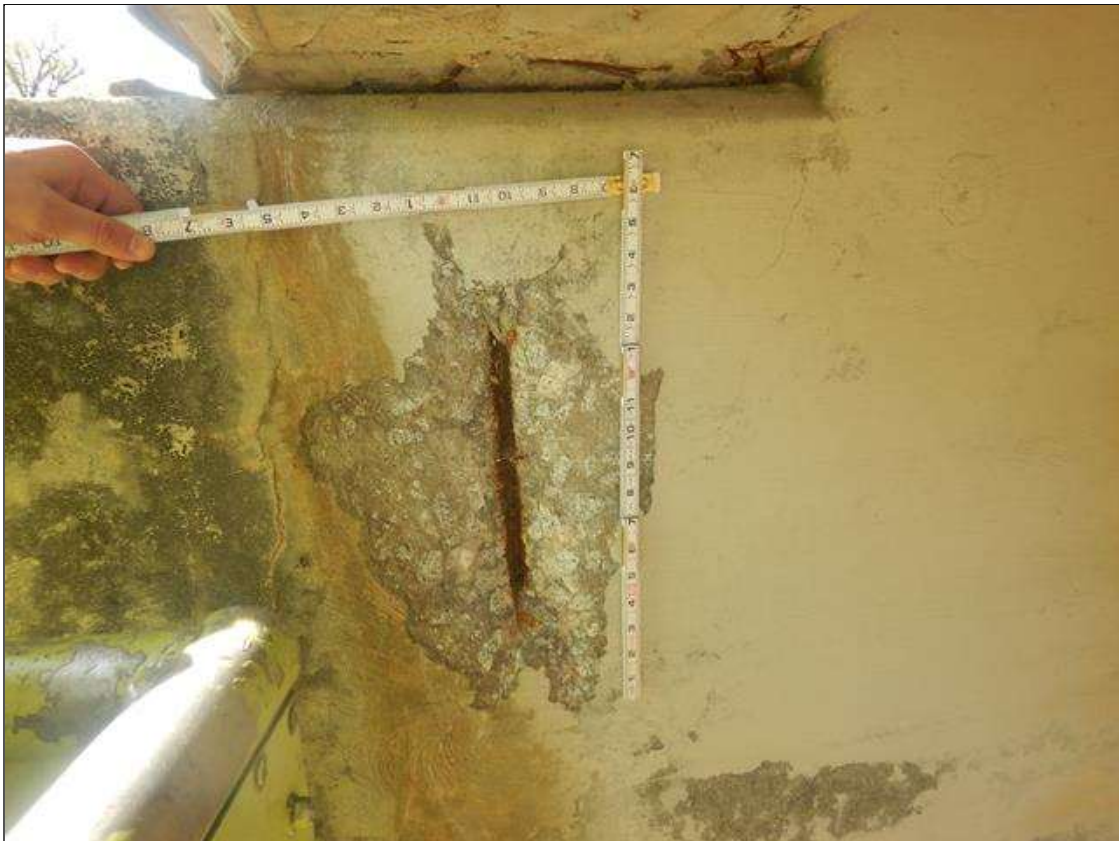
Bent 1 Cap 1: 16" HIGH X 11" WIDE X 1" DEEP SPALL WITH EXPOSED REINFORCEMENT WITH NO MEASURABLE SECTION LOSS EAST FACE UNDER BEAM 4
