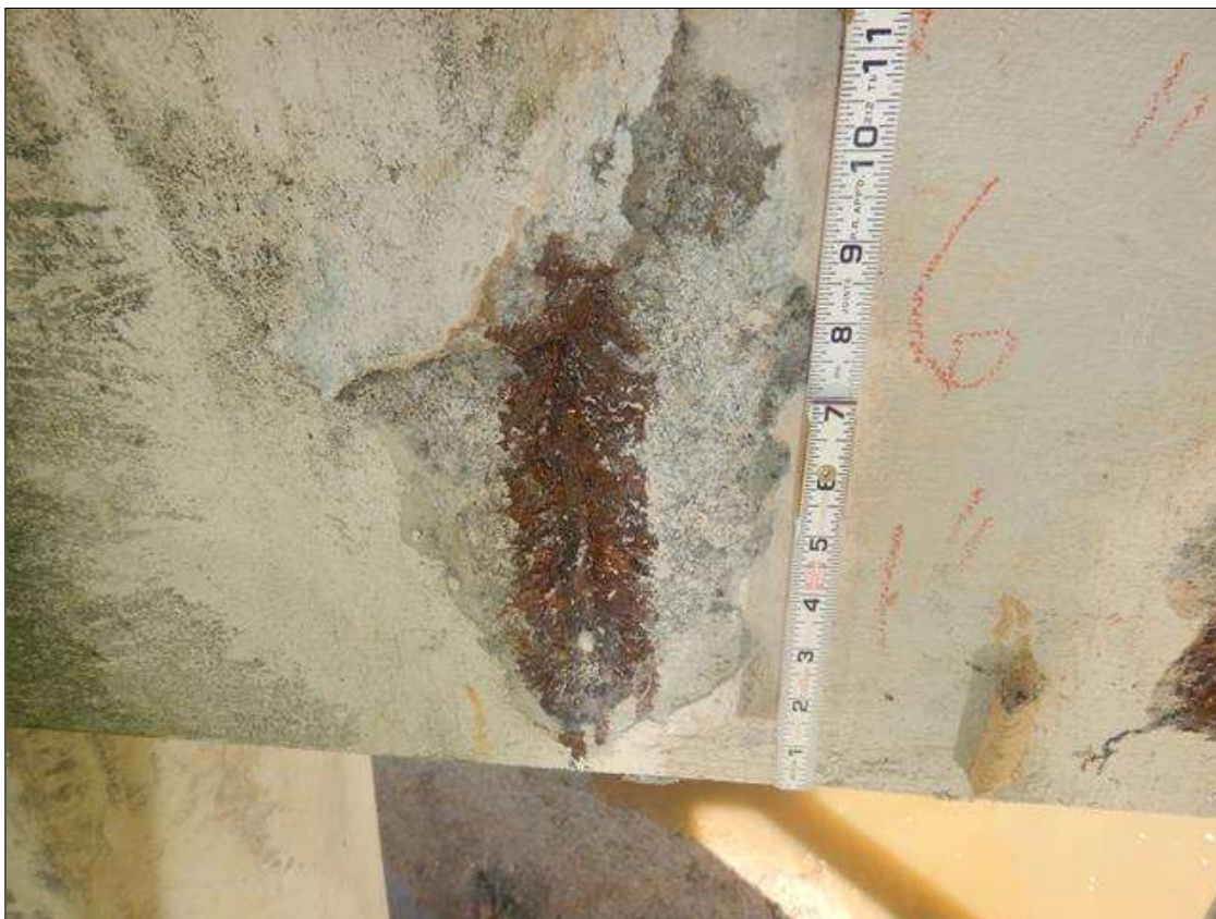
Bent 3 Cap 1: 1' HIGH X 6" WIDE X 1" DEEP SPALL WITH EXPOSED REINFORCING, NO MEASURABLE SECTION LOSS, AT BOTTOM OF WEST FACE BELOW BAY 1
