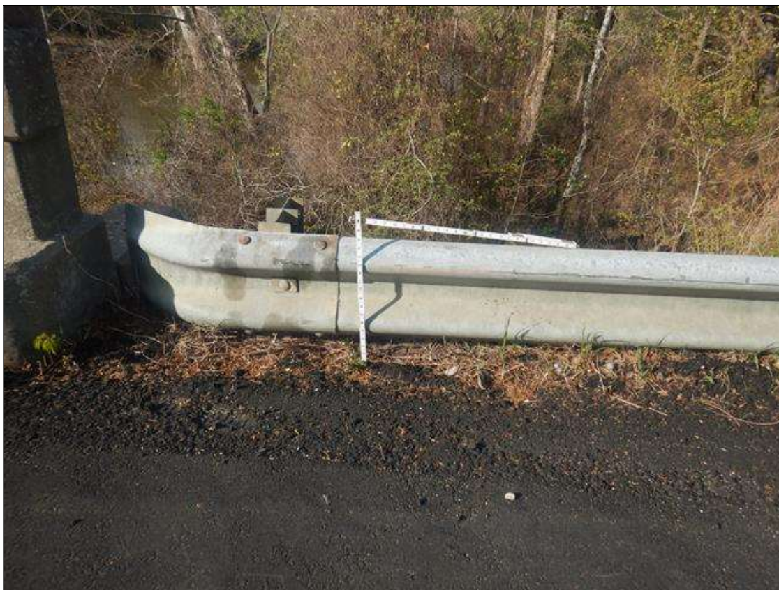
PAR: NORTHEAST GUARDRAIL IS SITTING ON GROUND, 14" HIGH CREATING A POTENTIAL SAFETY HAZARD
