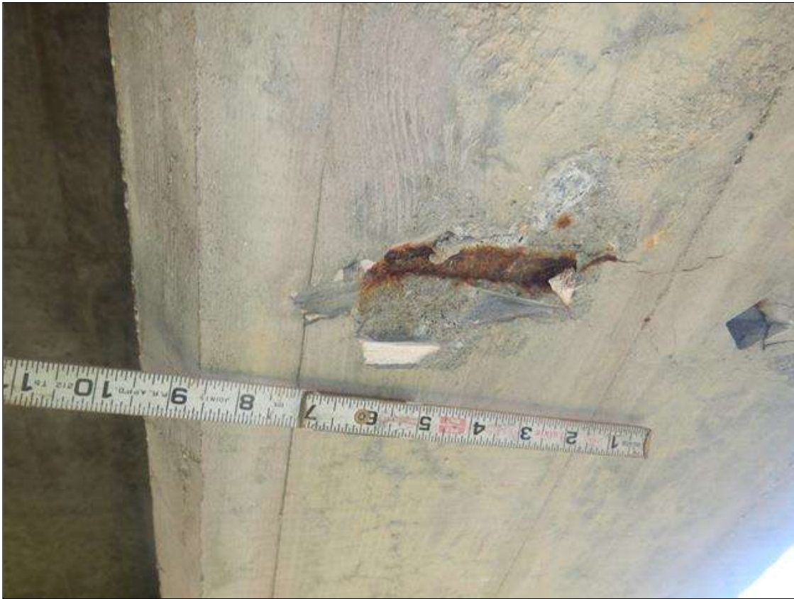
Span 10 Beam 1: 3" LONG X 4" WIDE X 1/2" DEEP SPALL WITH EXPOSED REINFORCEMENT IN BOTTOM FACE, LOCATED AT MIDSPAN. NO MEASURABLE SECTION LOSS IN EXPOSED REINFORCEMENT.
