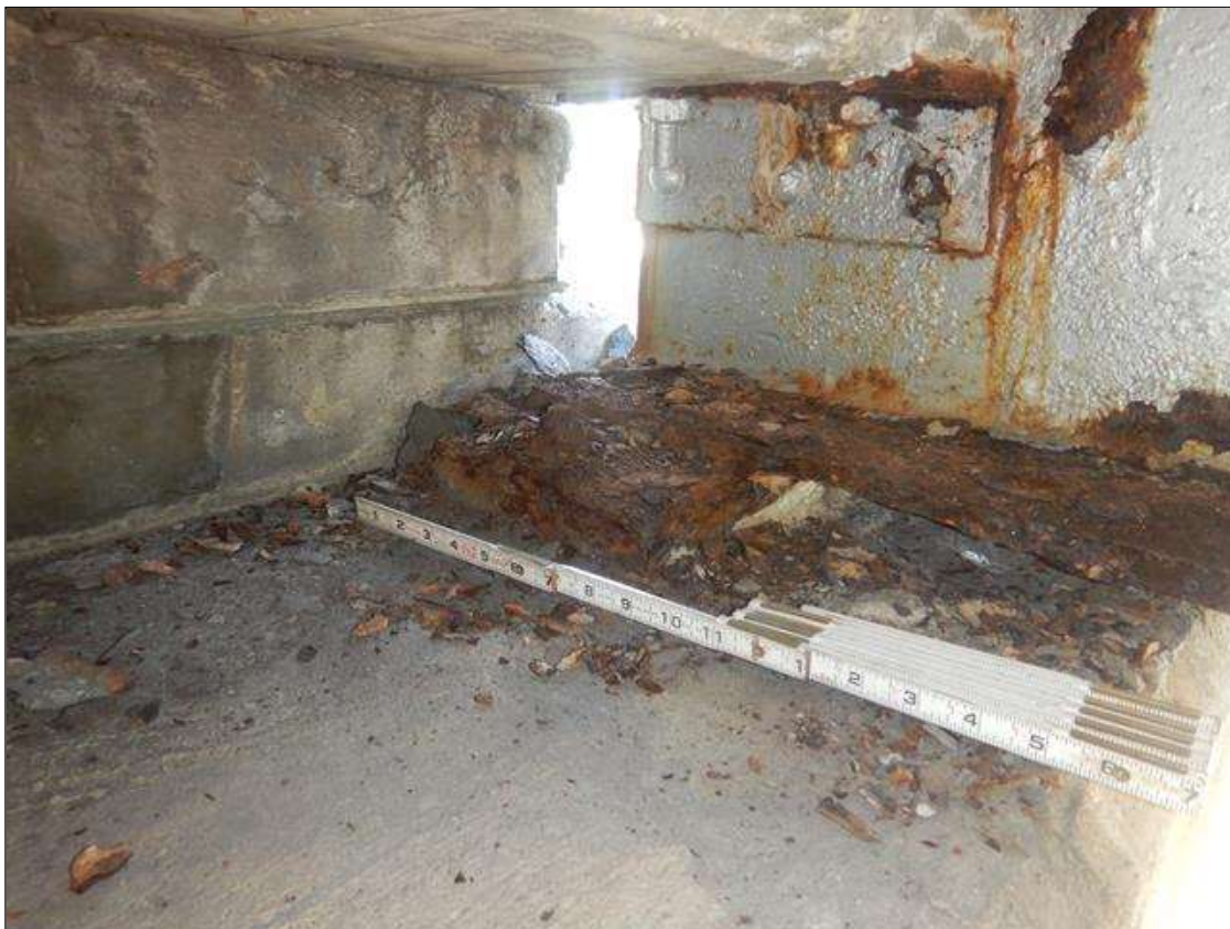
Span 6 Beam 5 - Far Bearing: CORROSION WITH MINOR DELAMINATION
