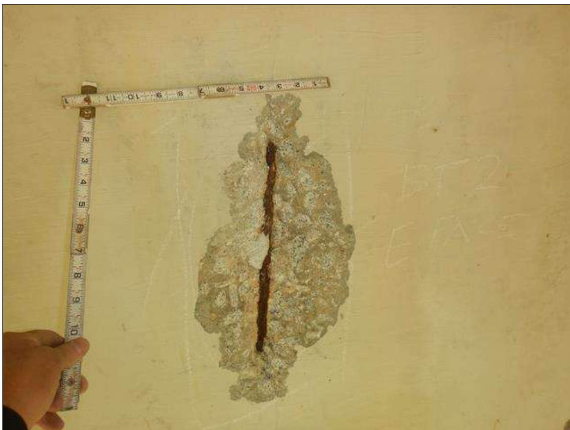
Bent 2 Cap 1: 1'-6" HIGH X 9" WIDE X 1" DEEP SPALL ON EAST FACE BELOW BAY 2 WITH EXPOSED REINFORCING, NO MEASURABLE SECTION LOSS
