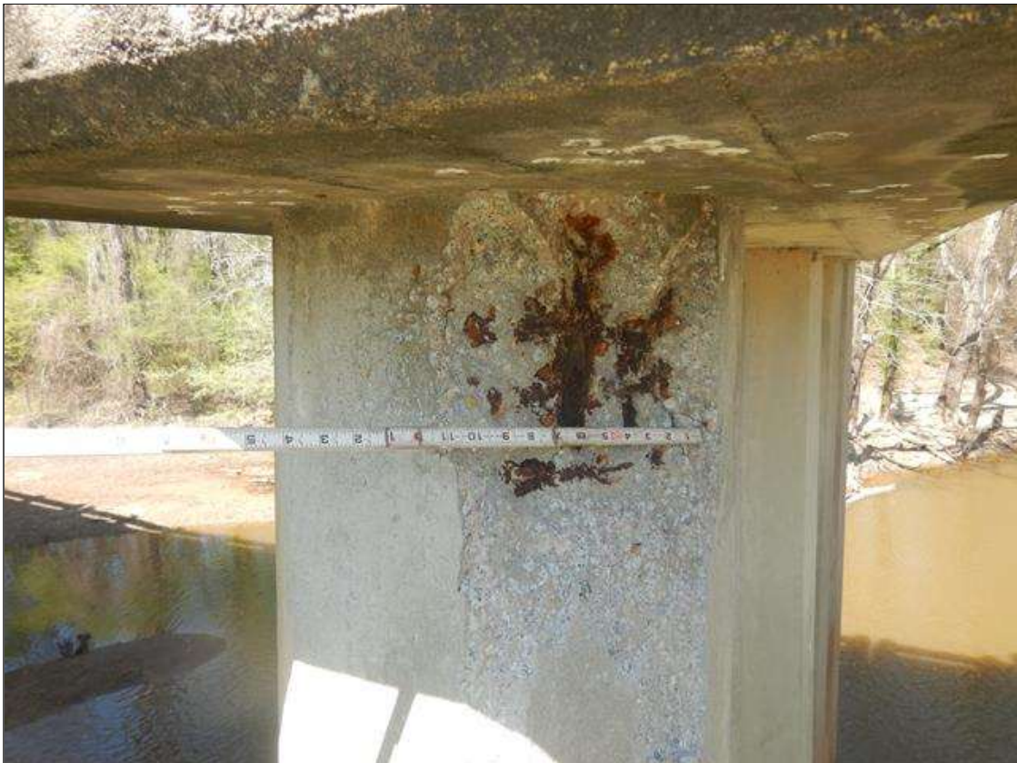
Bent 4 Pile 5: PAR: 2' HIGH X 11" WIDE X UP TO 2" DEEP SPALL WITH EXPOSED REINFORCEMENT IN SOUTHEAST FACE BELOW CAP
