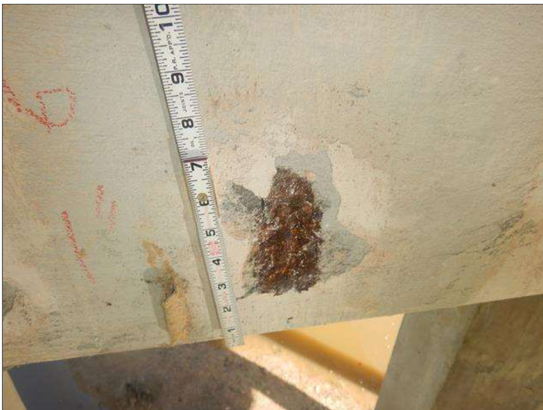
Bent 3 Cap 1: 6" HIGH X 4" WIDE X 1" DEEP SPALL WITH EXPOSED REINFORCING, NO MEASURABLE SECTION LOSS, AT BOTTOM OF WEST FACE BELOW BAY 1
