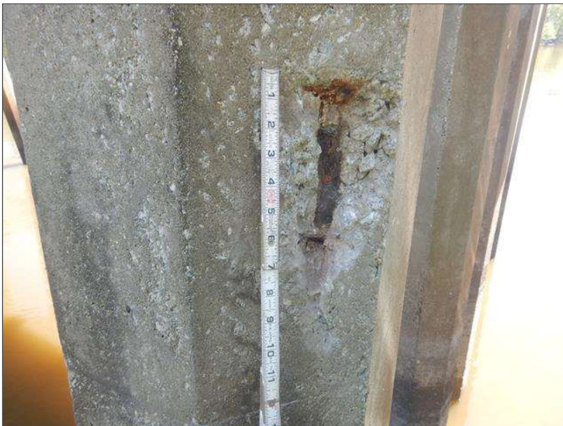
Bent 4 Pile 1: PAR: 10" HIGH X 6" WIDE X 2" DEEP SPALL WITH EXPOSED REINFORCEMENT WITH NO MEASURABLE SECTION LOSS AT NORTHWEST CORNER, MID HEIGHT
