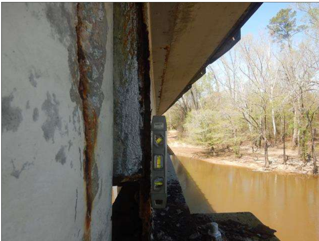
Span 6 Beam 1: PAR: UP TO 1'-6" LONG AREA OF DISTORTION IN THE WEB AT BOTH ENDS OF BEAM. WEB IS BOWED TO THE NORTH UP TO 1/2"
