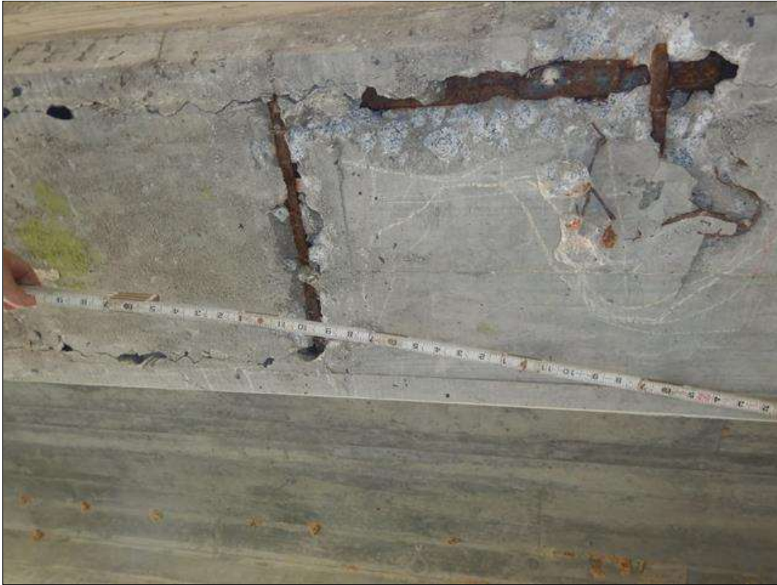
Span 10 Beam 3: PAR: 5' LONG X 18" WIDE AREA OF SPALLS WITH EXPOSED REINFORCEMENT AND UP TO 1/16" WIDE LONGITUDINAL CRACKS, STARTING 6' FROM END BENT 2 ON UNDERSIDE OF BEAM. SPALL SIZES VARY FROM 3" LONG X 6" WIDE X 1" DEEP TO 1'-6" LONG X 1' WIDE X 1 1/4" DEEP
