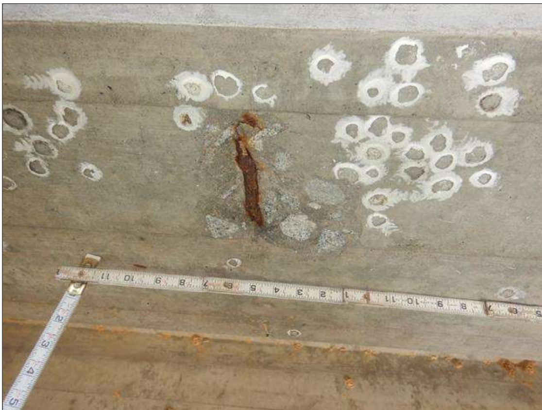
Span 7 Beam 4: (2) 7" LONG X 3" WIDE X 3/4" IN DEEP SPALL IN BOTTOM FACE WITH EXPOSED REINFORCEMENT, LOCATED AT 6 FT FROM BENT 7. NO MEASURABLE SECTION LOSS NOTED.
