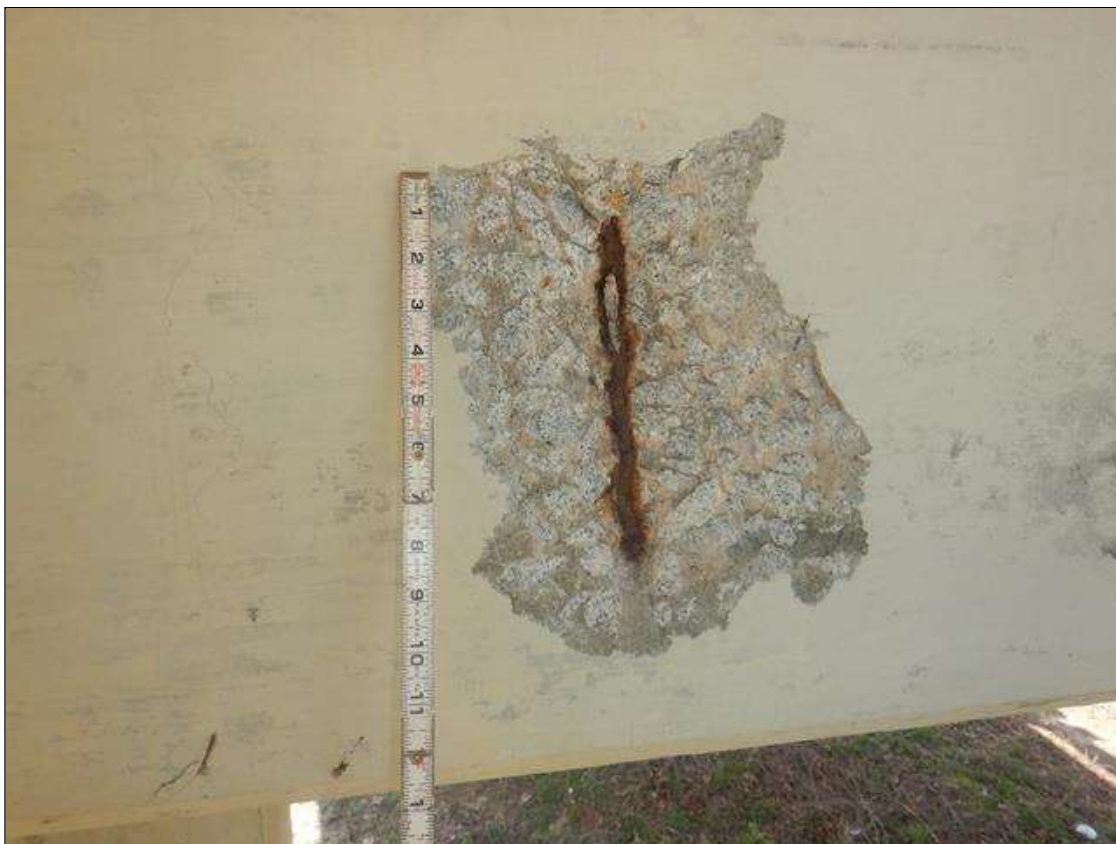
Bent 2 Cap 1: 1' HIGH X 9" WIDE X 1" DEEP SPALL ON EAST FACE BELOW BAY 1 WITH EXPOSED REINFORCING, NO MEASURABLE SECTION LOSS
