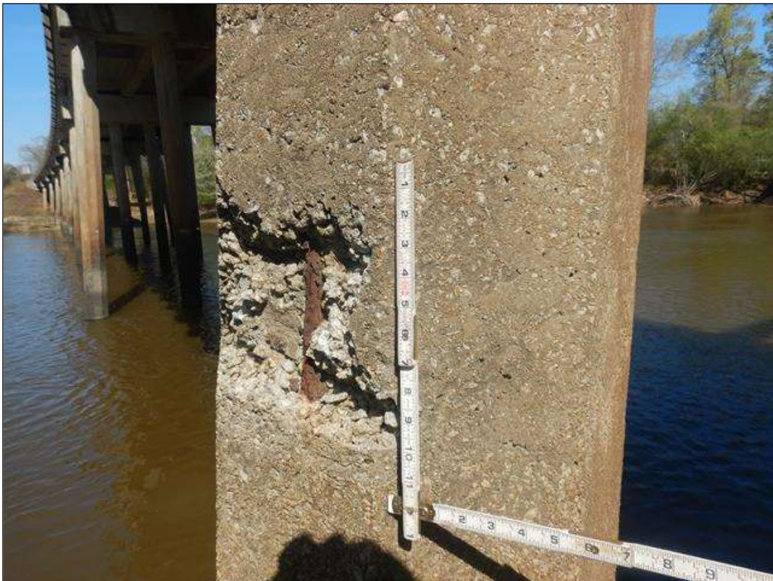
Bent 8 Pile 5: PAR: 7" HIGH X 1' WIDE X 2" DEEP SPALL WITH EXPOSED REINFORCEMENT WITH MINOR SECTION LOSS IN SOUTH FACE, AT 12' FROM WATER LEVEL.
