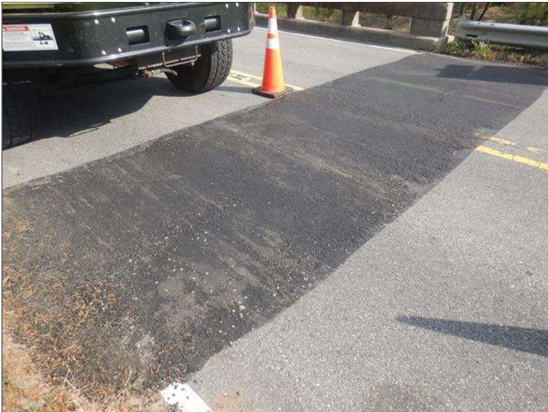
7' LONG X FULL WIDTH WEDGE PATCH HAS BEEN ADDED TO THE WEST APPROACH ROADWAY SINCE PREVIOUS INSPECTION
