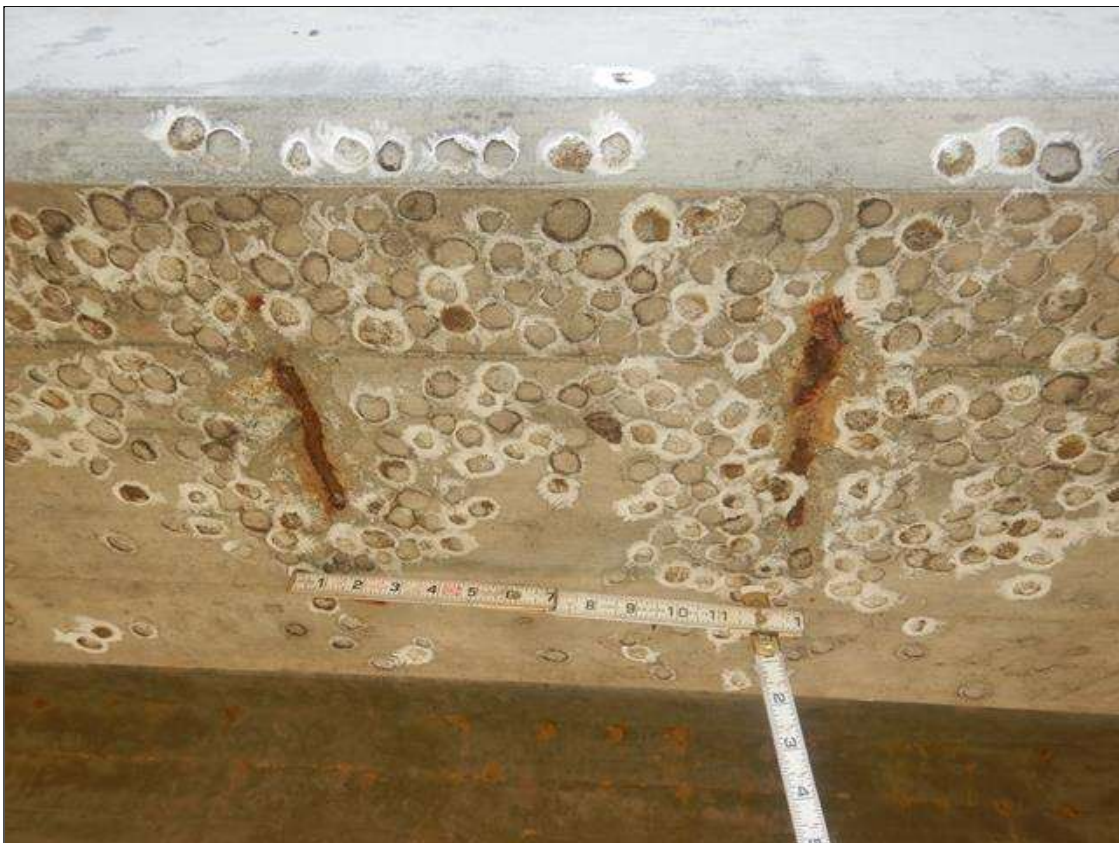
Span 7 Beam 1: (2) UP TO 7 IN WIDE X 2 IN LONG X 3/4 IN DEEP SPALLS WITH EXPOSED REINFORCEMENT IN BOTTOM FACE, LOCATED AT 7 FT FROM BENT 6
