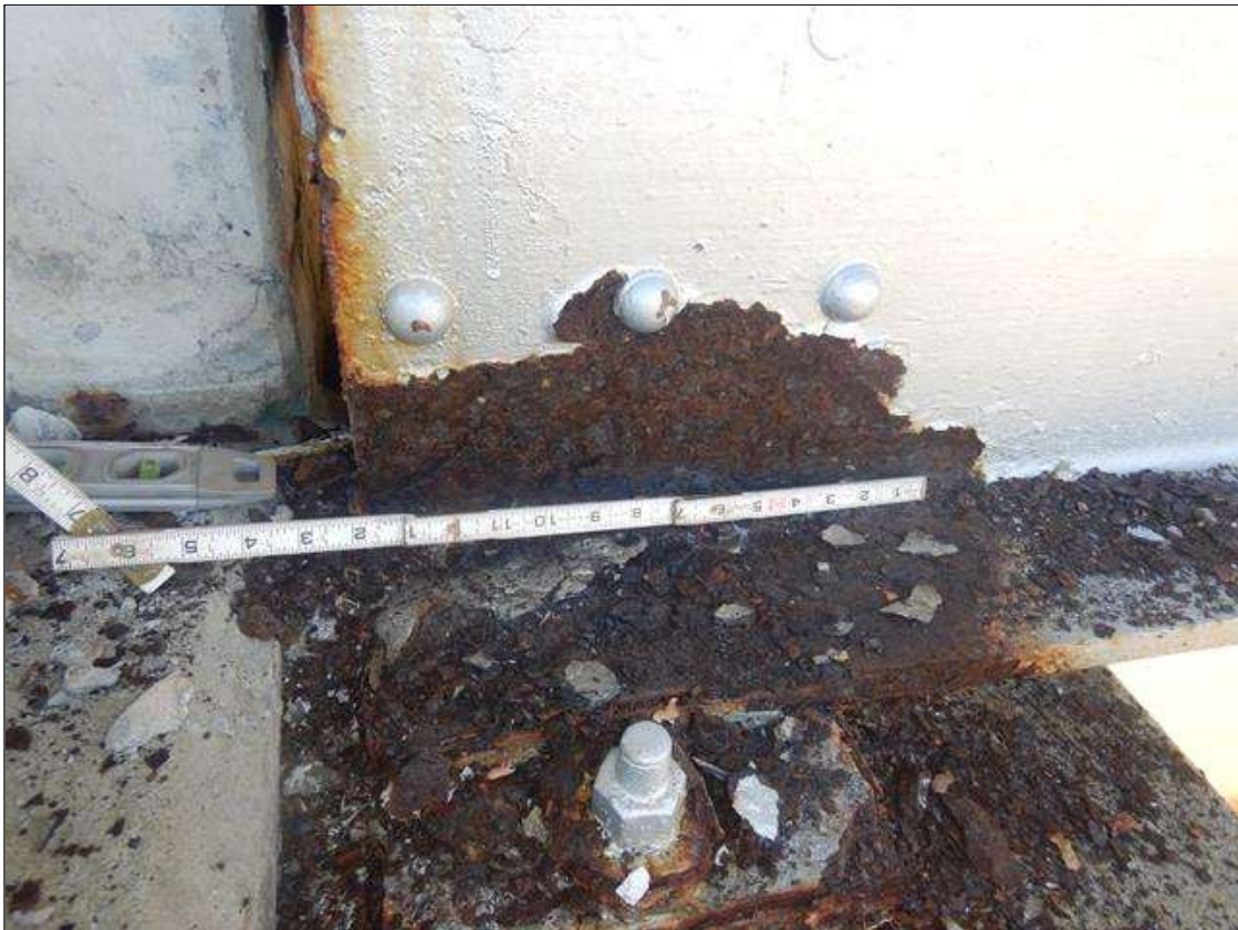
Span 6 Beam 1: 1' LONG X 6" HIGH AREA OF CORROSION WITH SECTION LOSS ON BOTTOM OF WEB AT BENT 6, 1/2" REMAINING
