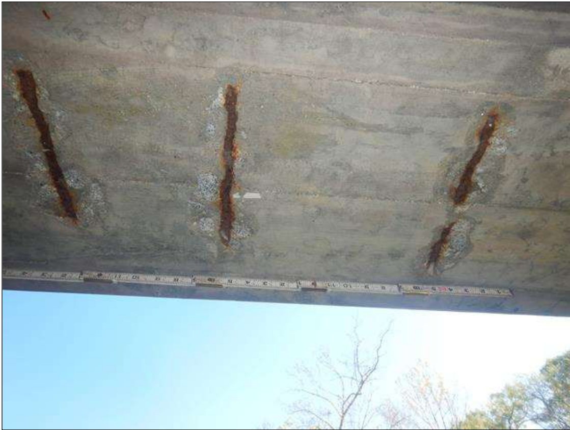
Span 10 Beam 1: THREE (3) 11" WIDE X 3" LONG X 1/2" DEEP SPALLS WITH EXPOSED REINFORCEMENT IN BOTTOM FACE, LOCATED AT 6 FT FROM BENT 9. NO MEASURABLE SECTION LOSS IN EXPOSED REINFORCEMENT.
