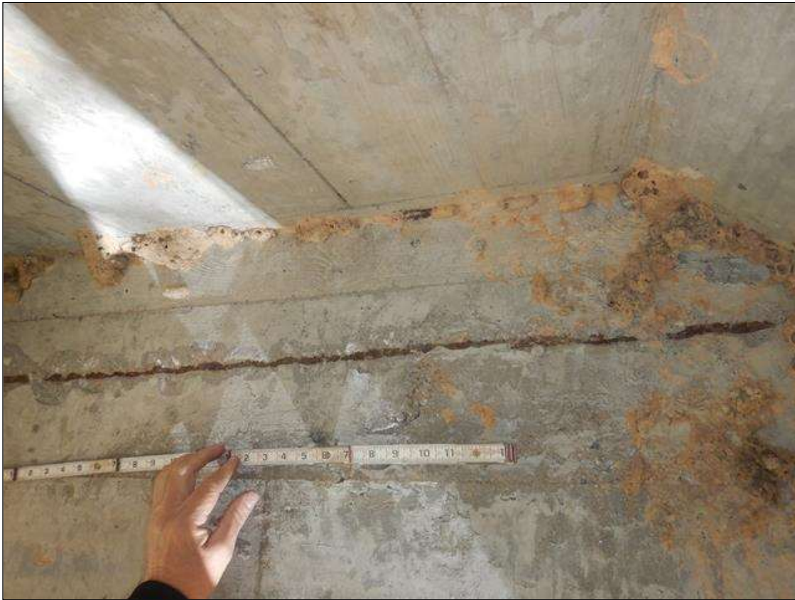
5 FT LONG X 2.5 IN HIGH X 1/2 IN DEEP SPALL WITH EXPOSED REINFORCEMENT IN INTERMEDIATE DIAPHRAGM SPAN 4 BAY 1, WEST FACE. NO MEASURABLE SECTION LOSS IN EXPOSED REINFORCEMENT
