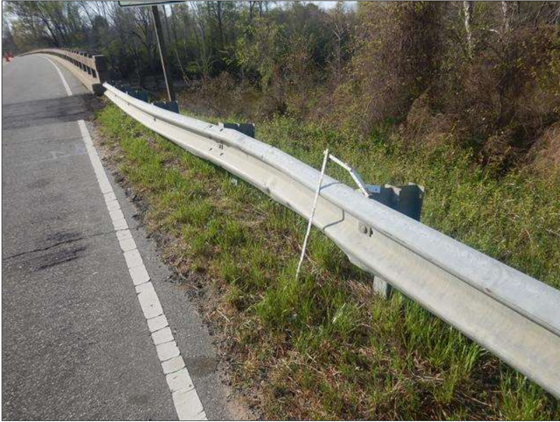
PAR: MODERATE AREA OF IMPACT DAMAGE ON NORTHWEST GUARDRAIL STARTING APPROXIMATELY 30' FROM EAST APPROACH, POSTS 5, 6, AND 7 ARE LEANING AND POSTS 6 AND 7 ARE TWISTED
