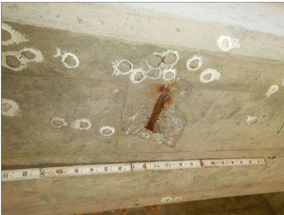
Span 7 Beam 4: (2) 7" LONG X 3" WIDE X 3/4" IN DEEP SPALL IN BOTTOM FACE WITH EXPOSED REINFORCEMENT, LOCATED AT 6 FT FROM BENT 7. NO MEASURABLE SECTION LOSS NOTED.
