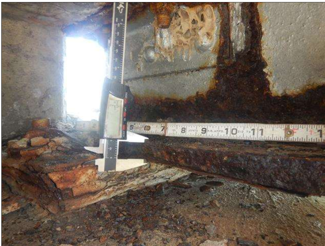
Span 6 Beam 1: PAR: 1' LONG X FULL WIDTH AREA OF CORROSION WITH 1/4" SECTION LOSS ON BOTTOM FLANGE AT BENT 5, 3/4" REMAINING
