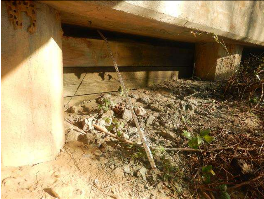
End bent 2 Abutment: PAR: FULL LENGTH X UP TO 1'-8" HIGH X FULL DEPTH VOID UNDER CAP WITH ALL PILES EXPOSED. THERE IS A TIMBER BACKWALL IN PLACE BEHIND PILES 4-5. THERE IS NO RETAINING MEASURE IN PLACE TO HOLD BACK FILL FOR THE REMAINDER OF CAP LENGTH
