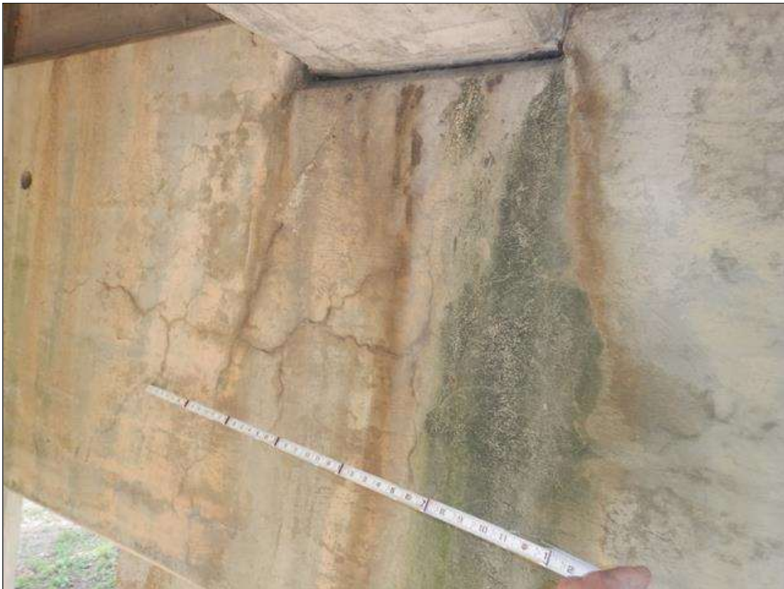
Bent 1 Cap 1: FULL HEIGHT AREA OF HAIRLINE MAP CRACKING WITH EFFLORESCENCE AND LEAKAGE STAINS IN WEST FACE, BELOW BAYS 2 AND 3
