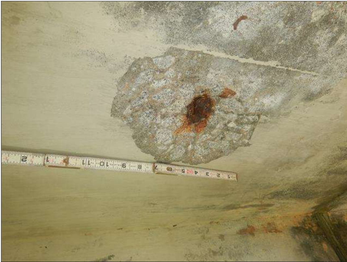
Span 7 Deck: 8" LONG X 6" WIDE X 1" DEEP SPALL IN RIGHT OVERHANG WITH EXPOSED REBAR, LOCATED OVER BENT 6 & 7. (OVER BENT 7 SHOWN)
