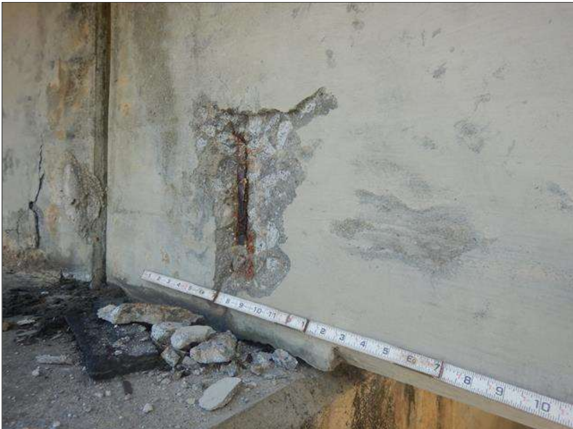
Span 9 Beam 4: 1' HIGH X 10" WIDE X 3/4 IN DEEP SPALL WITH EXPOSED REINFORCEMENT NO MEASURABLE SECTION LOSS IN SOUTH FACE AT BENT 8
