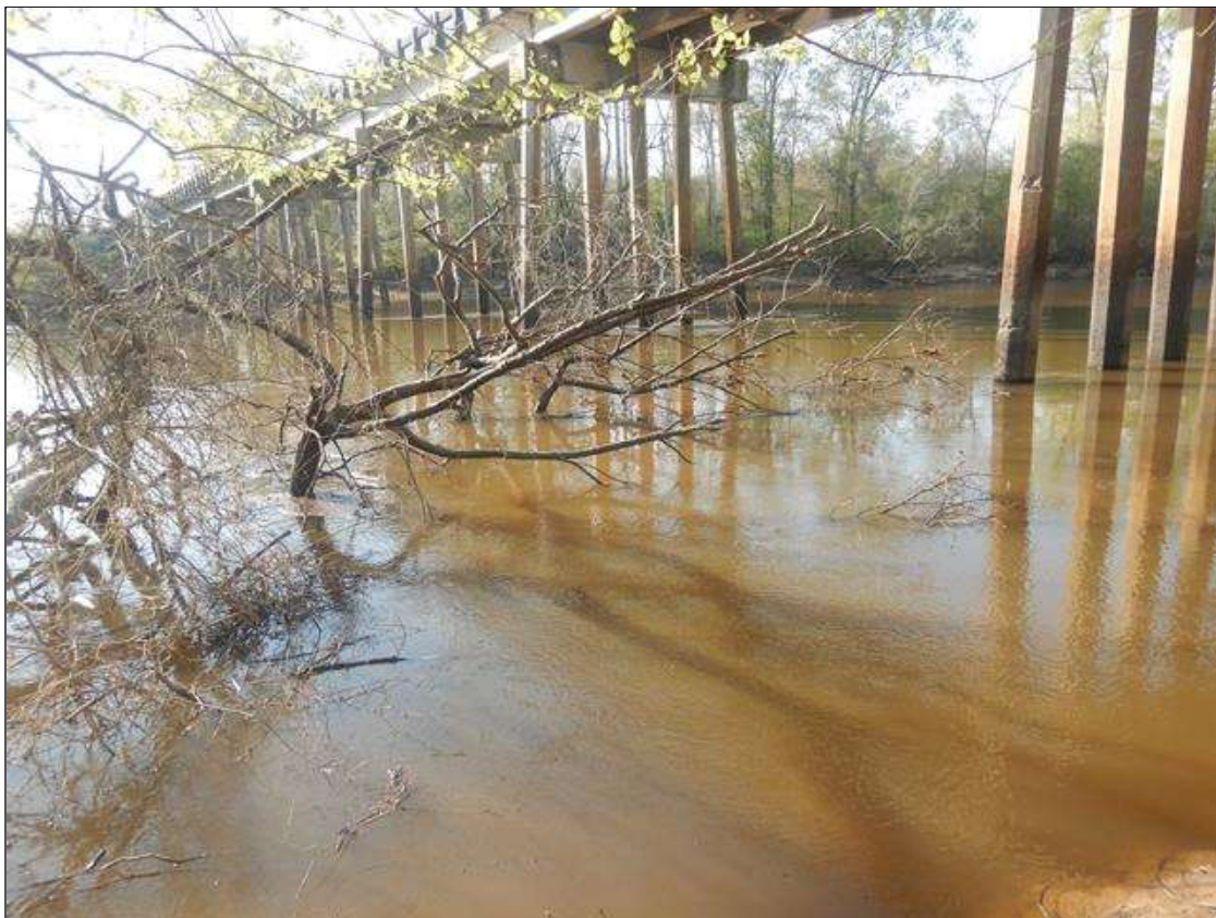
PAR: AREA OF FALLEN TREES AND DRIFT UPSTREAM OF BENTS 7 AND 8 CREATING A PARTIAL BLOCKAGE
