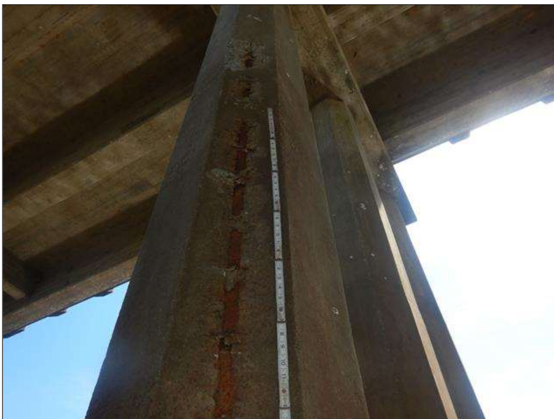
Bent 4 Pile 3: PAR: 9' HIGH X 8" WIDE X 1" DEEP SPALL AND DELAMINATION WITH EXPOSED REINFORCEMENT AND NO MEASURABLE SECTION LOSS AT NORTHWEST CORNER.
