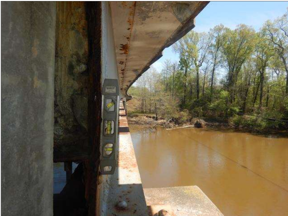
Span 6 Beam 5: PAR: UP TO 6" LONG AREA OF DISTORTION IN WEB AT BOTH ENDS OF BEAM. WEB IS BOWED TO THE SOUTH UP TO 1/2"
