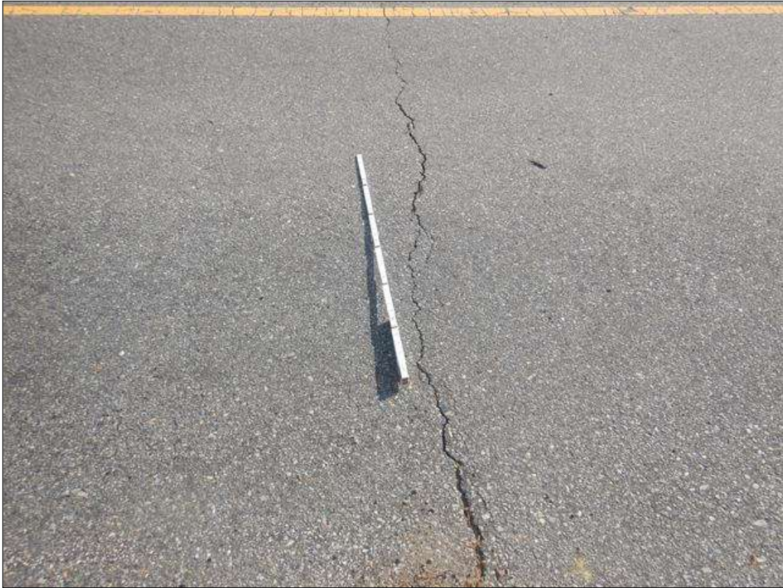
Span 1 Wearing Surface: UP TO 3/16" WIDE X FULL DECK WIDTH CRACK OVER BENT 1, CRACK EXPANDS TO 1 1/2" WIDE IN SHOULDERS
