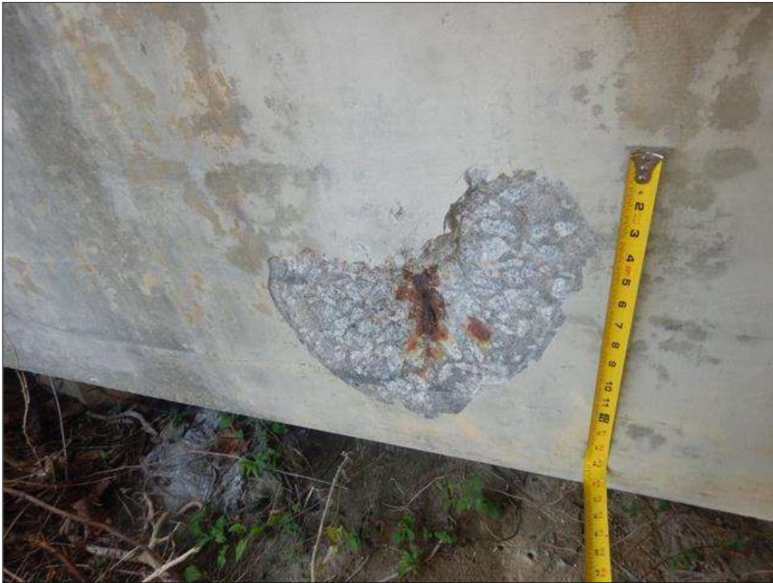
End bent 1 Cap 1: UP TO 15" WIDE X 12" HIGH X 1" DEEP SPALL WITH EXPOSED REINFORCEMENT UNDER BEAM 4 WITH NO MEASURABLE SECTION LOSS
