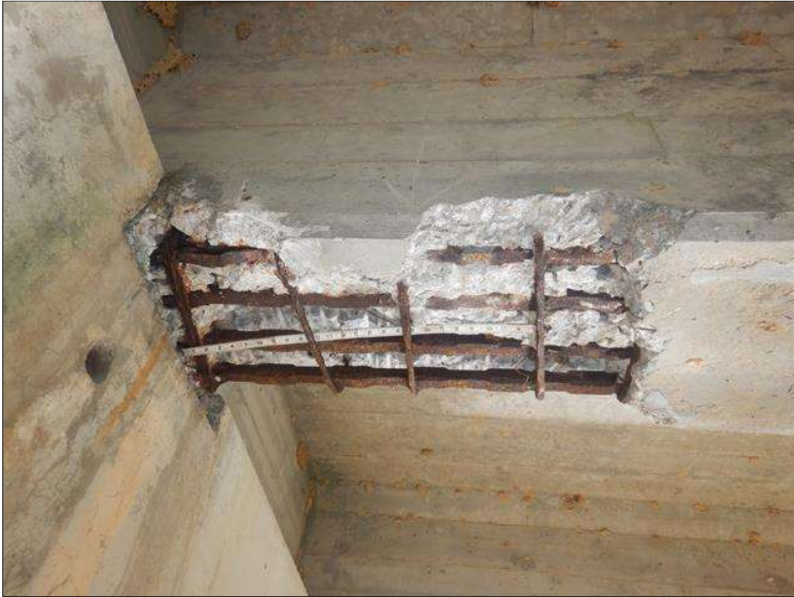
Span 3 Beam 3: PAR: 3'-8" LONG X 18" WIDE X UP TO 5" DEEP SPALL WITH EXPOSED REINFORCEMENT IN BOTTOM FLANGE AT BENT 3, EXTENDING 13" HIGH ON THE SOUTH FACE AND 4" HIGH ON THE NORTH FACE. FOUR LONGITUDINAL BARS AND 6 STIRRUPS EXPOSED WITH NO MEASURABLE SECTION LOSS IN LONGITUDINAL BARS AND 60% AVG SECTION REMAINING IN STIRRUPS.
