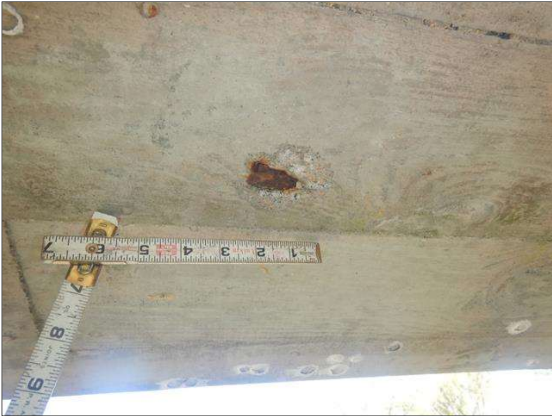
Span 9 Beam 1: 2" DIAMETER X 3/16" DEEP SPALL WITH EXPOSED REINFORCEMENT IN BOTTOM FACE, LOCATED AT 15 FT FROM BENT 9. NO MEASURABLE SECTION LOSS IN EXPOSED REINFORCEMENT.
