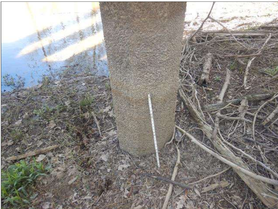
Bent 2 Pile 1: EXPOSED AGGREGATE AND ABRASION FOR 5 FT STARTING AT GROUND LEVEL.
