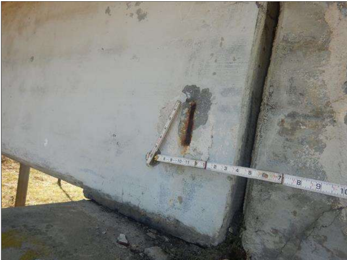
Span 9 Beam 1: 3" WIDE X 6" HIGH X 1/2" DEEP SPALL WITH EXPOSED REINFORCEMENT IN NORTH FACE, LOCATED OVER BENT 8. NO MEASURABLE SECTION LOSS IN EXPOSED REINFORCEMENT.
