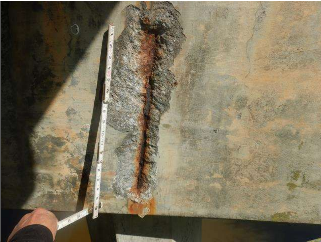
Bent 3 Cap 1: 1'-8" HIGH X 6" WIDE X 1" DEEP SPALL WITH EXPOSED REINFORCEMENT WITH NO MEASURABLE SECTION LOSS IN WEST FACE, BELOW BEAM 4.
