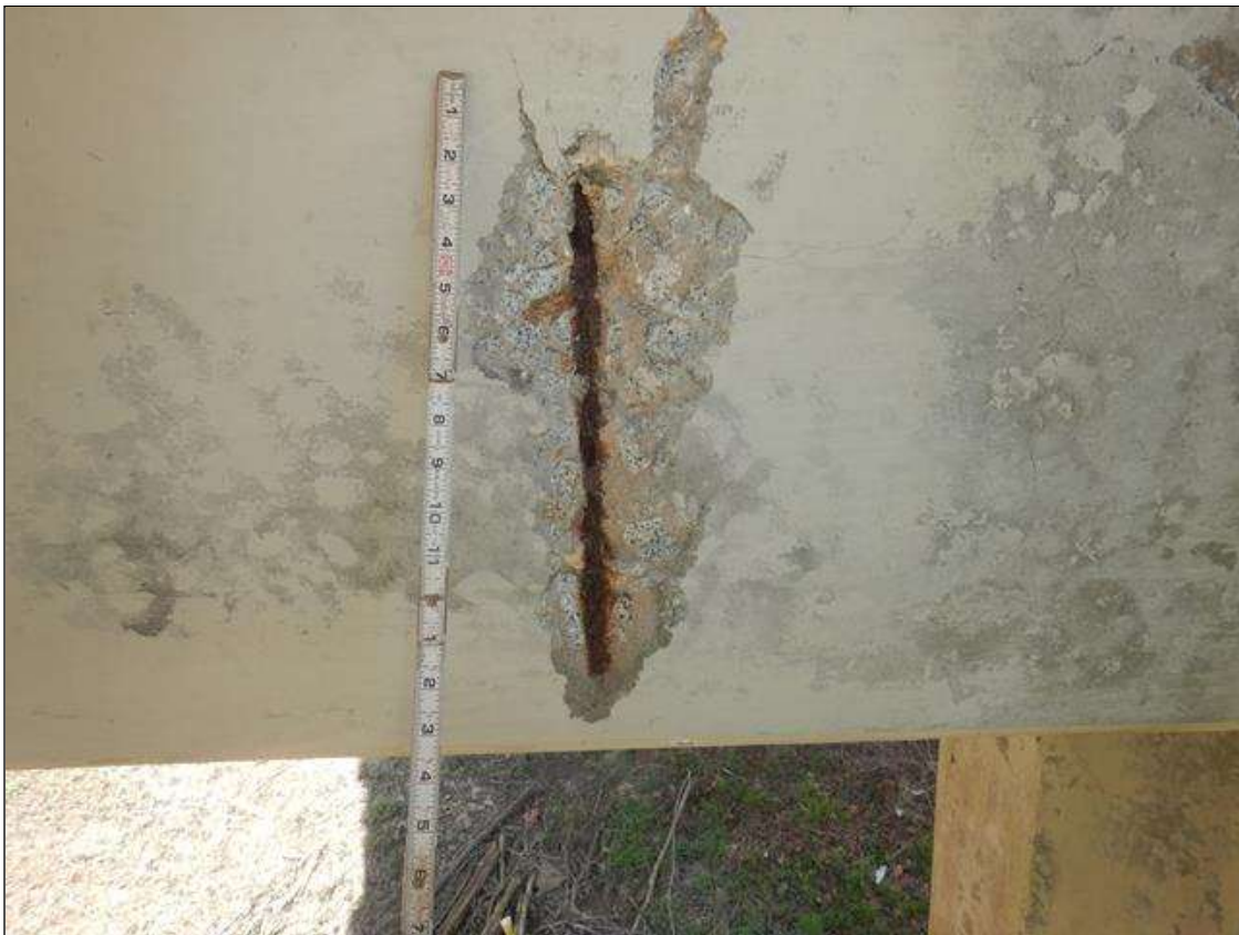
Bent 2 Cap 1: 17" HIGH X 5" WIDE X 1" DEEP SPALL WITH EXPOSED REINFORCEMENT WITH NO MEASURABLE SECTION LOSS ON EAST FACE BELOW BEAM 1
