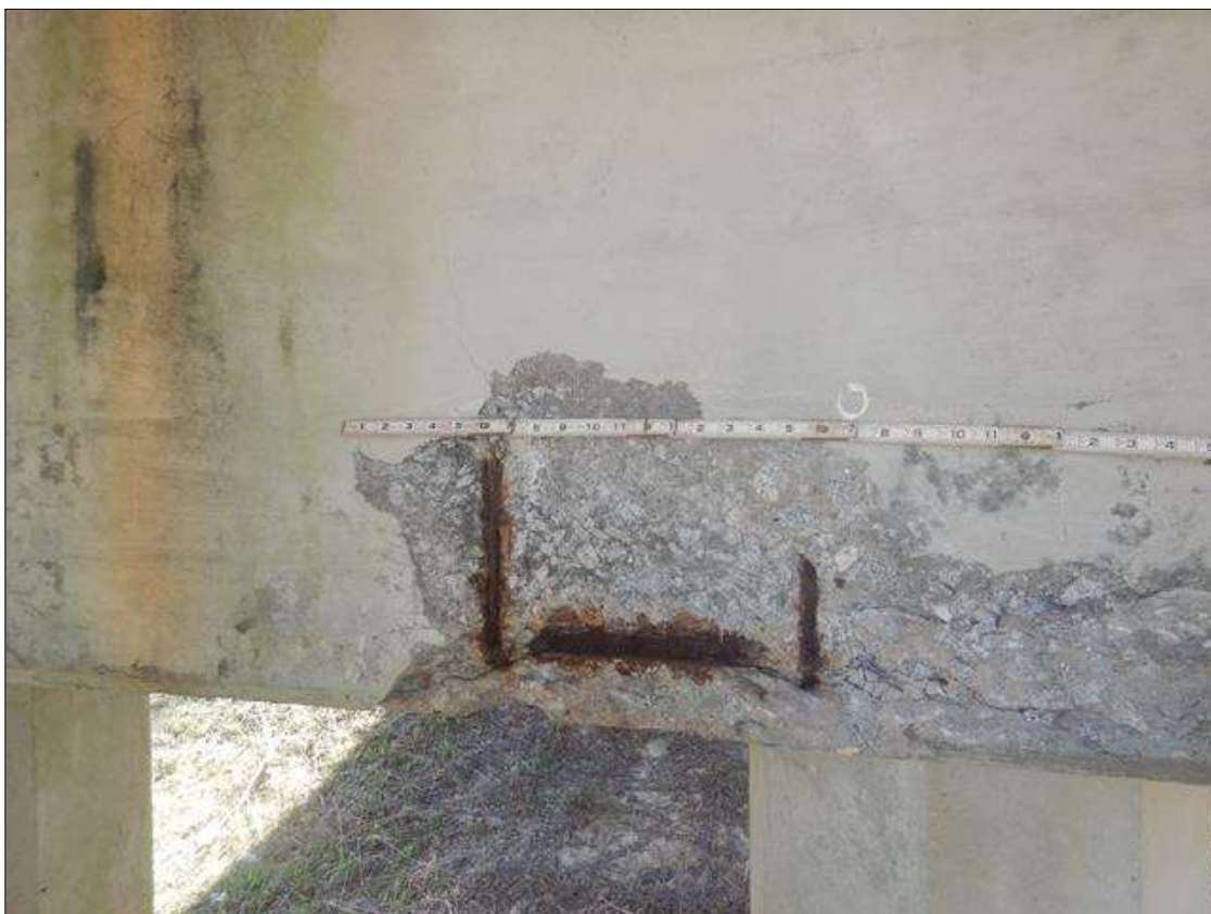
Bent 9 Cap 1: 3'-6" WIDE X 1'-2" HIGH X UP TO 3" DEEP SPALL WITH EXPOSED REINFORCEMENT ON WEST FACE ABOVE PILE 4, NO MEASURABLE SECTION LOSS
