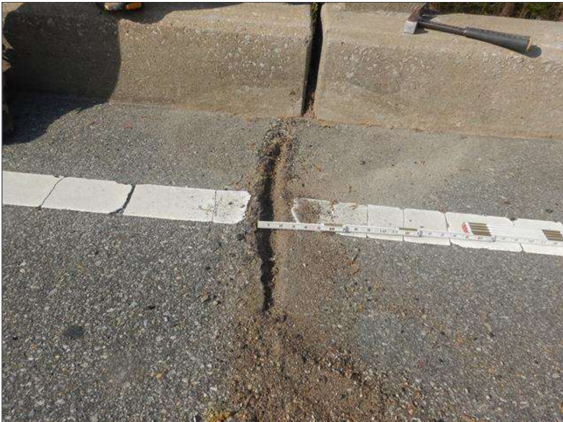
Span 1 Wearing Surface: UP TO 3/16" WIDE X FULL DECK WIDTH CRACK OVER BENT 1, CRACK EXPANDS TO 1 1/2" WIDE IN SHOULDERS
