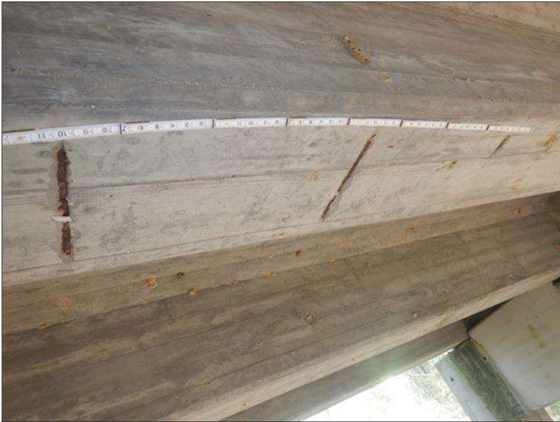
Span 1 Beam 3: (3) 11" LONG X 1" WIDE X 1/4" DEEP SPALLS WITH EXPOSED REINFORCEMENT WITH NO MEASURABLE SECTION LOSS IN BOTTOM FLANGE BETWEEN INTERIOR DIAPHRAGM AND BENT 1.
