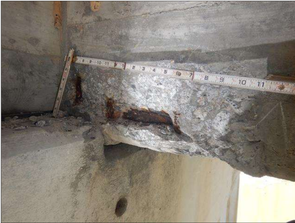
Span 5 Beam 3: PAR: 18" LONG X 7" HIGH X 1 1/2" DEEP SPALL WITH EXPOSED REINFORCING IN SOUTH FACE, STARTING AT BENT 4
