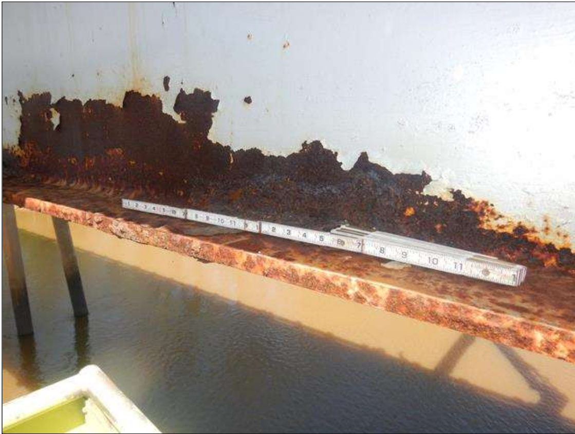
Span 6 Beam 5: CORROSION WITH MINOR DELAMINATION IN TOP AND BOTTOM FLANGES, AND BOTTOM 6 IN OF WEB FOR 11 FT LONG, STARTING AT 6 FT FROM BENT 6. NO MEASURABLE SECTION LOSS NOTED
