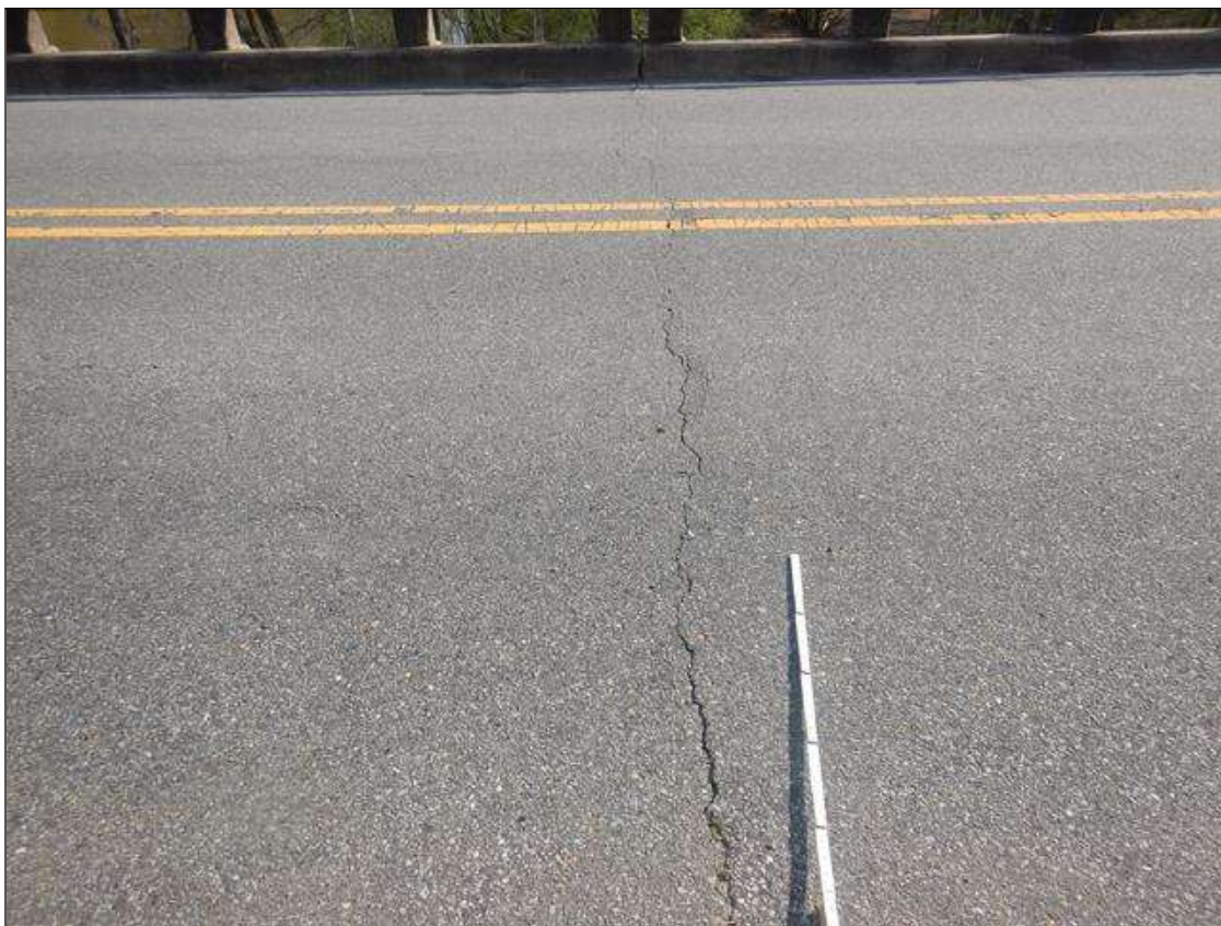
Span 2 Wearing Surface: UP TO 1/8" WIDE X FULL DECK WIDTH CRACK OVER BENT 2, CRACK EXPANDS TO 1 1/4" WIDE IN SHOULDERS
