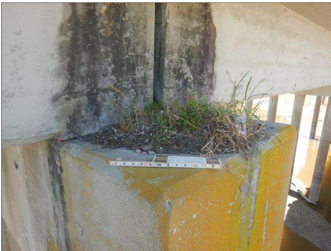
HEAVY VEGETATION GROWTH ON TOP FACE OF BENT 4 CAP BELOW NORTH OVERHANG
