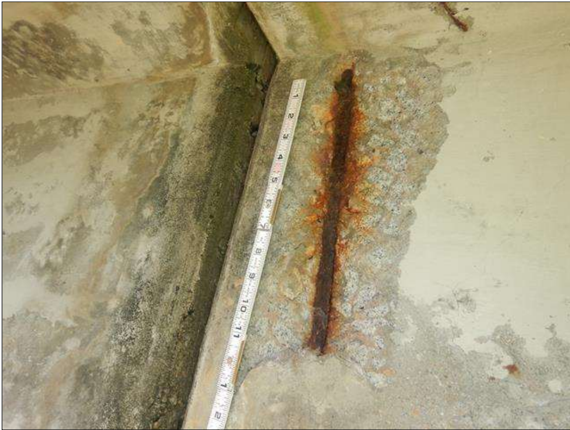
Span 2 Beam 4: PAR: 11" HIGH X 6" WIDE X 1" DEEP SPALL WITH EXPOSED REINFORCEMENT WITH MINOR SECTION LOSS (1/16") IN SOUTH FACE AT BENT 1.
