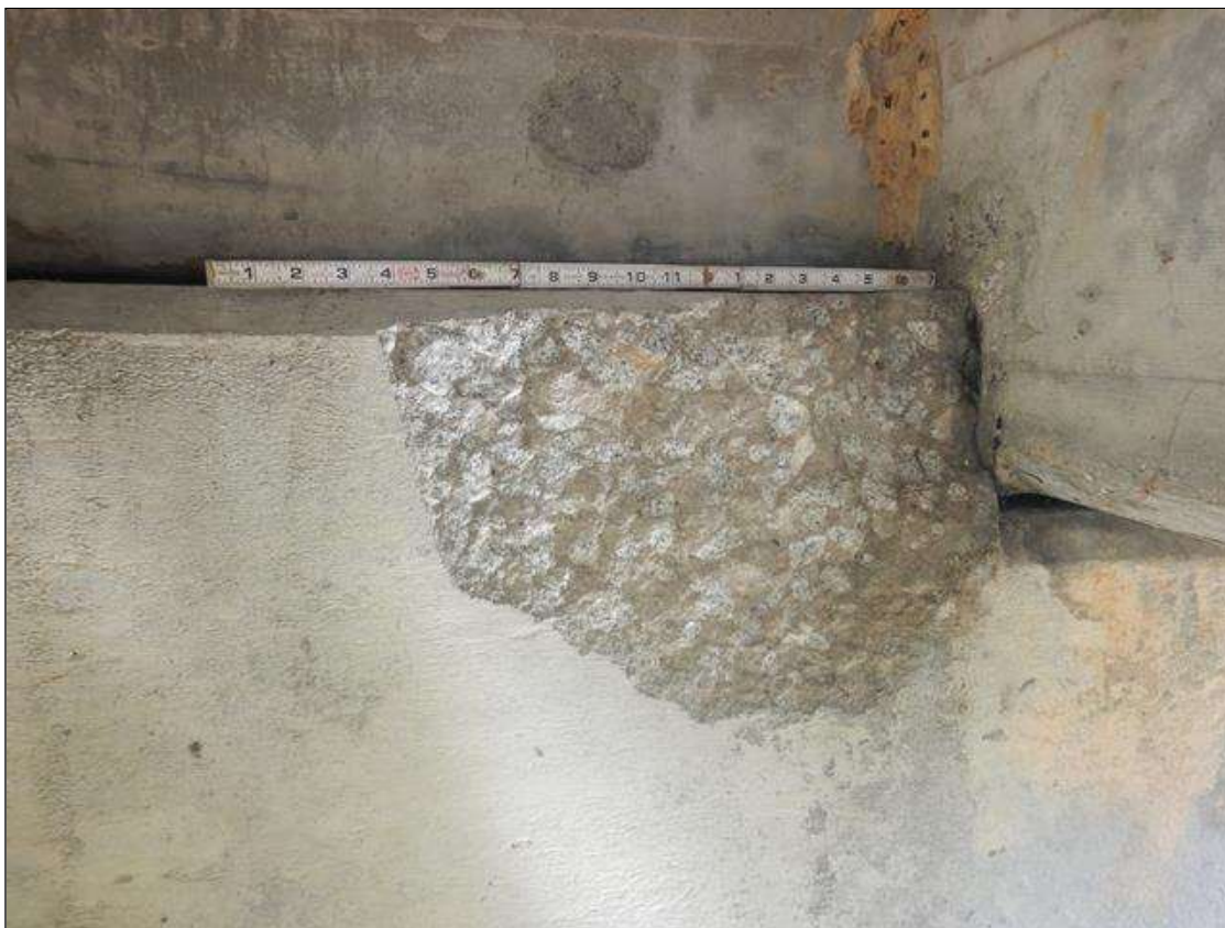
Bent 4 Cap 1: 1'-4" LONG X 10" HIGH X UP TO 2" DEEP SPALL IN TOP OF CAP, WEST FACE, BAY 3.
