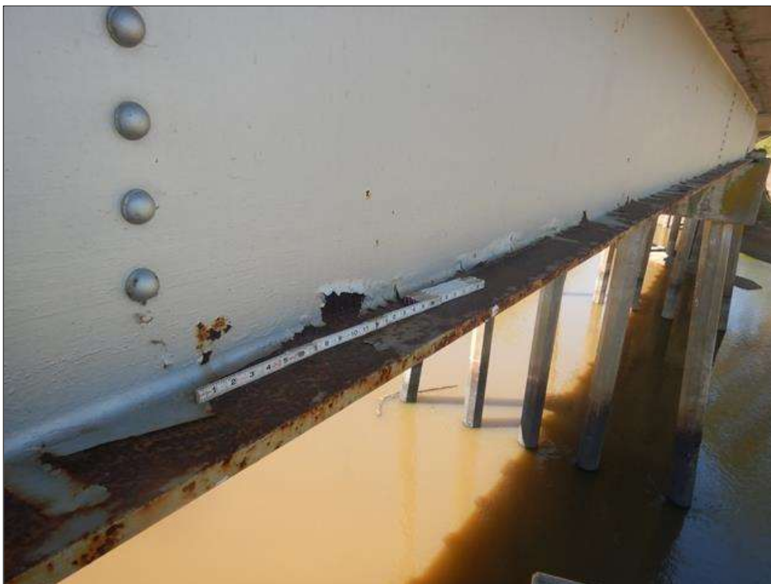
Span 6 Beam 1: MINOR SURFACE CORROSION ON TOP OF BOTTOM FLANGE AND WEB, FOR FULL LENGTH EXCEPT FOR BEAM ENDS.
