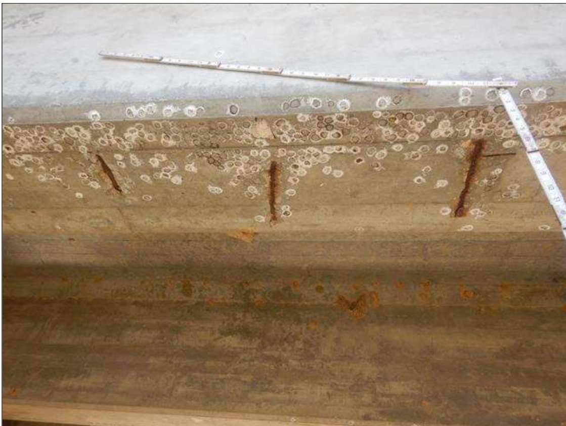
Span 7 Beam 1: (3) UP TO 10" WIDE X 1 1/2" LONG X 1/2" DEEP SPALLS WITH EXPOSED REINFORCEMENT AND NO MEASURABLE SECTION LOSS IN BOTTOM FACE, STARTING AT 11 1/2' FROM BENT 7
