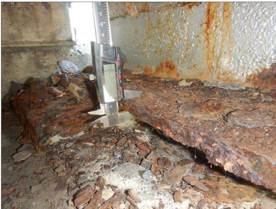
Span 6 Beam 5: PAR: 7" LONG X 2" WIDE AREA OF CORROSION WITH 3/8" SECTION LOSS ON NORTH SIDE OF BOTTOM FLANGE AT BENT 6. 5/8" REMAINING
