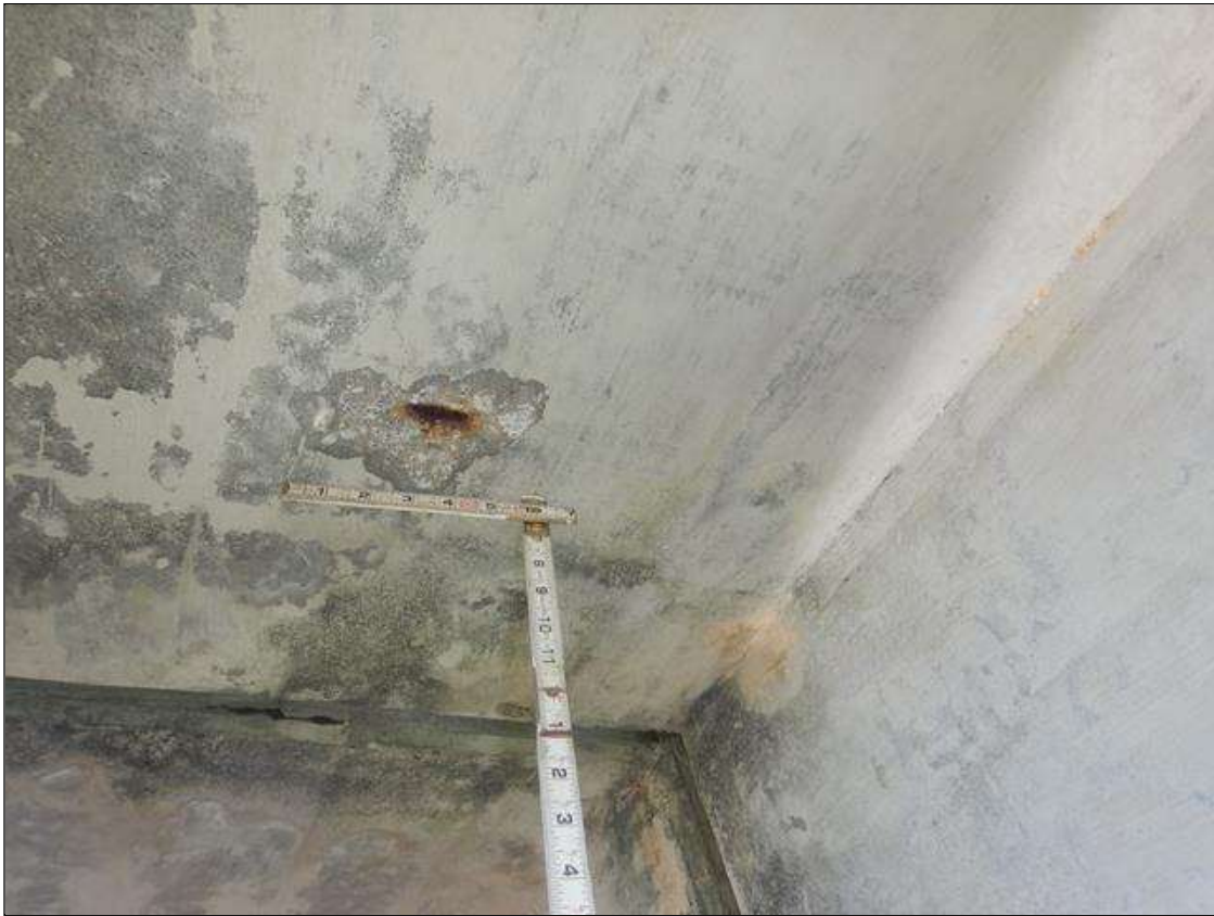
Span 9 Deck: 6" WIDE X 4" LONG X 1/2" DEEP SPALL WITH EXPOSED REBAR IN RIGHT OVERHANG AT BENT 8
