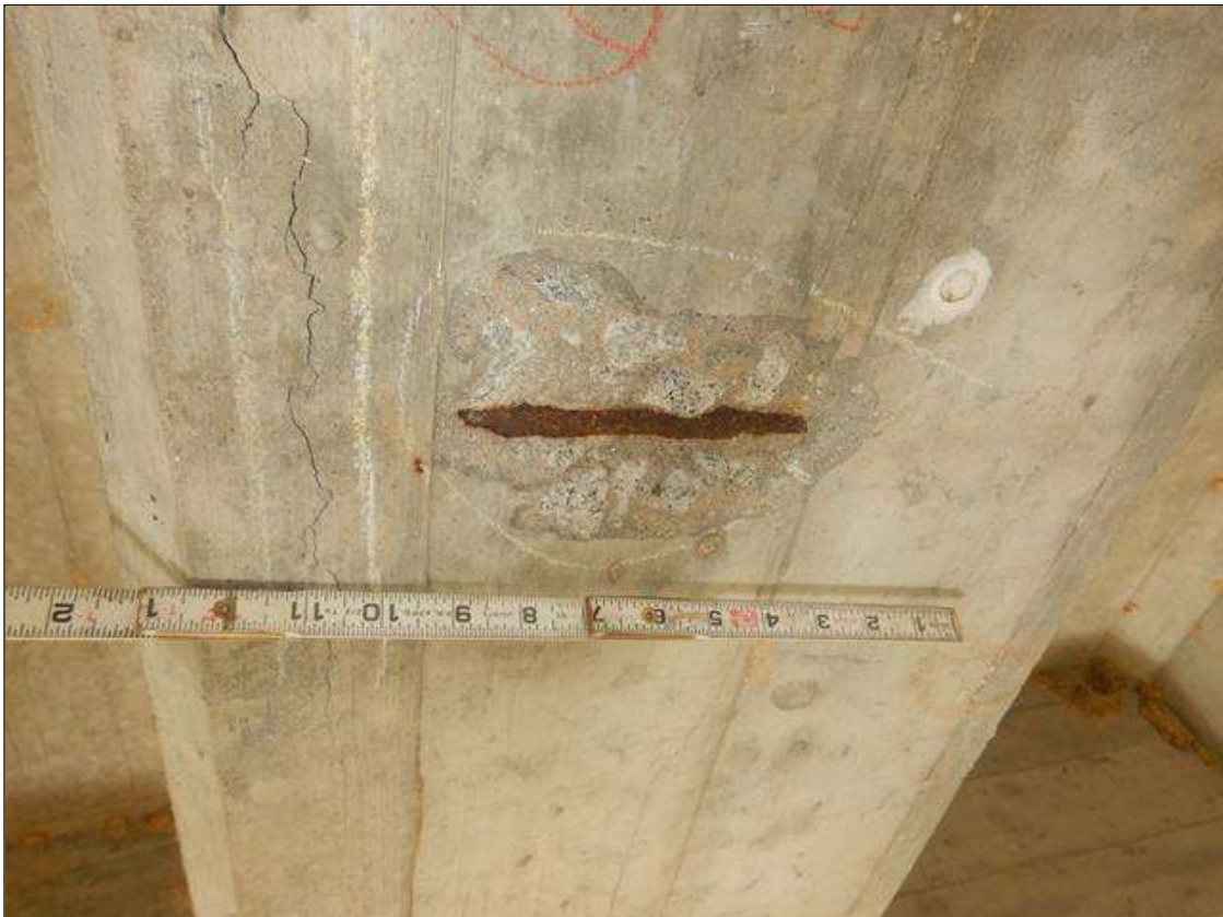
Span 4 Beam 3: (2) SPALLS WITH EXPOSED REINFORCEMENT IN BOTTOM FLANGE, 17' FROM BENT 4, UP TO 7" LONG X 4" WIDE X 1/2" DEEP. NO MEASURABLE SECTION LOSS IN EXPOSED REINFORCEMENT
