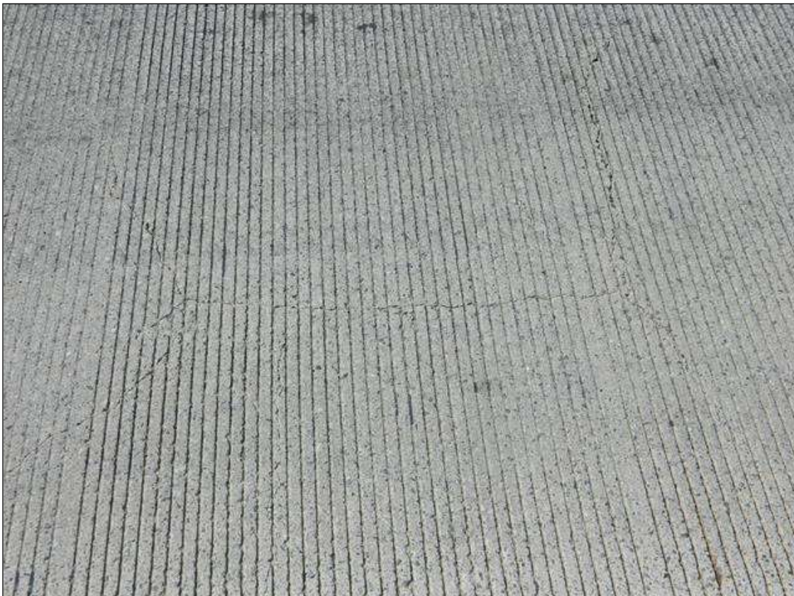
Span 3 Wearing Surface: MULTIPLE HAIRLINE CRACKS SCATTERED THROUGHOUT THE WEARING SURFACE.
