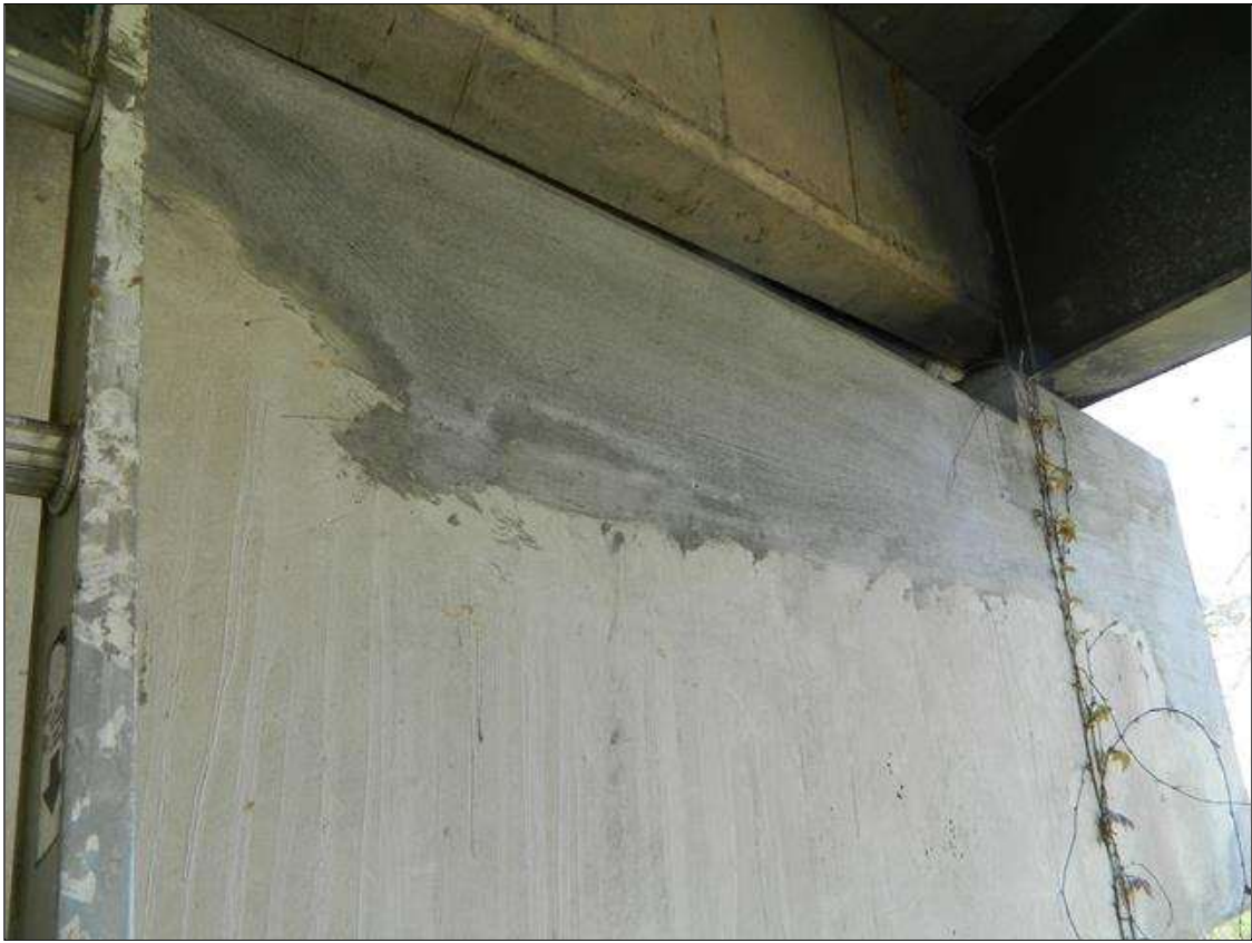
Bent 1 Cap 1: MULTIPLE PATCHED AREAS THAT ARE SOUND.
