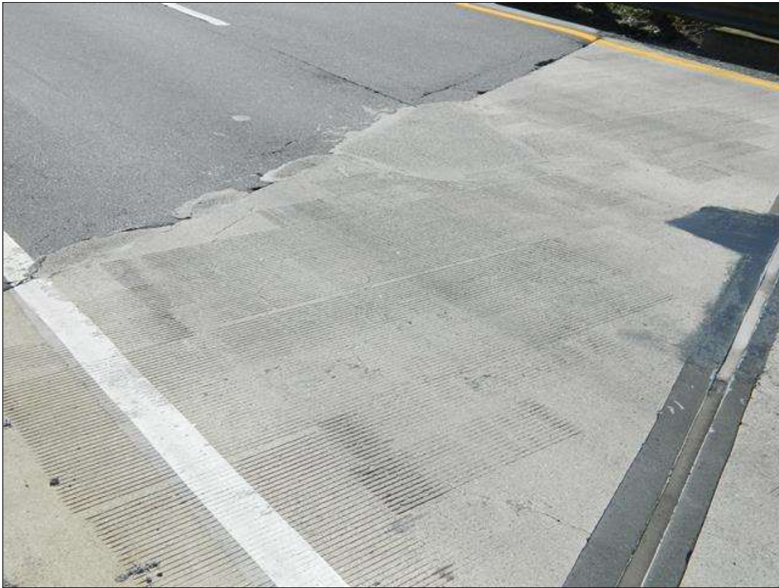
Approach 2: DIAGONAL AND LONGITUDINAL CRACKS THROUGHOUT
