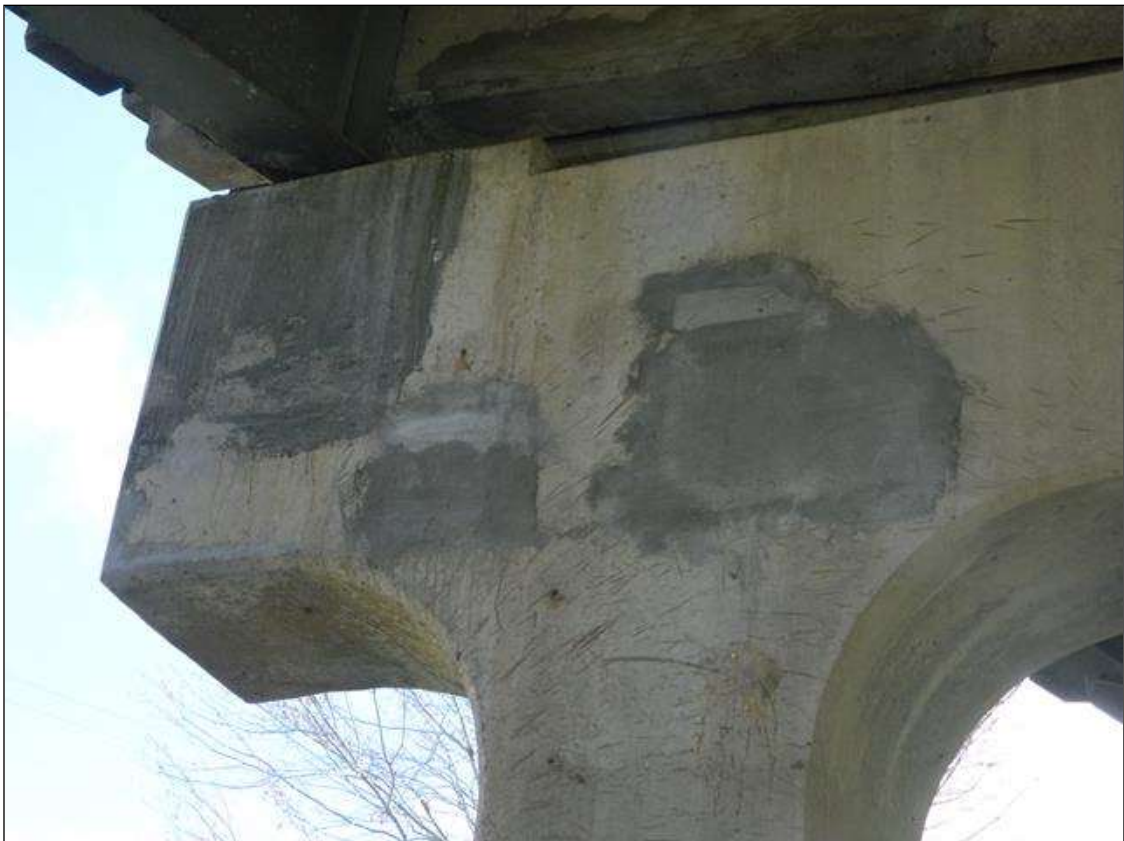
Bent 2 Cap 1: MULTIPLE SOUND PATCHED AREAS
