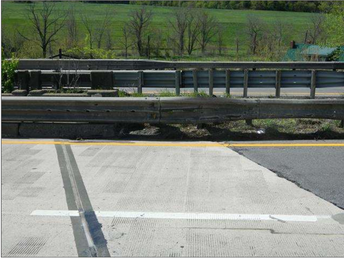
Span 1 Right Bridge Rail: 14' LONG SCRAPE DAMAGE AT THE NEAR END OF THE SPAN.
