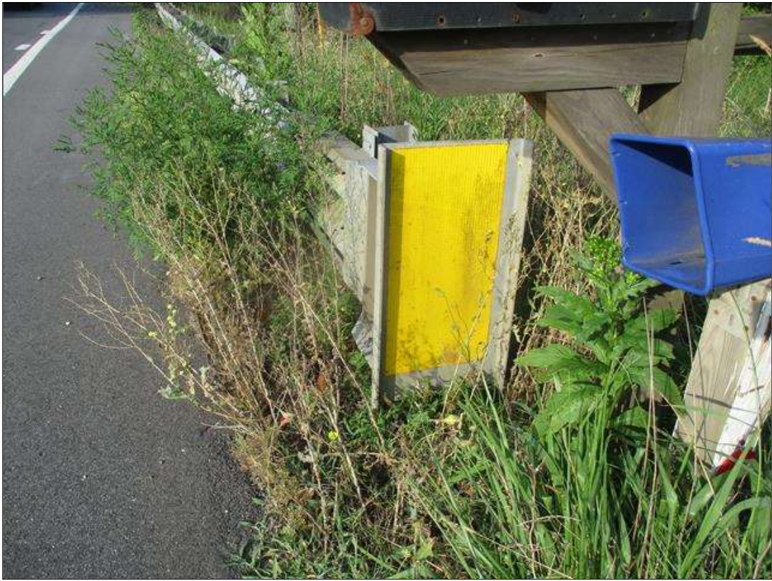
GUARDRAIL TERMINAL END
