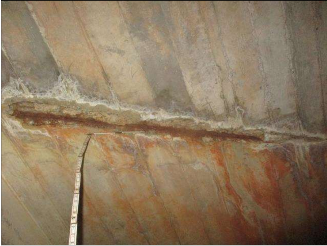
Span 1 Culvert Section 1: FULL WIDTH X 7 INCHES LONG X 3 INCHES DEEP SPALLED AREA WITH EXPOSED REINFORCEMENT AND EFFLORESCENCE IN THE TOP SLAB, 14 FEET FROM THE UPSTREAM END OF THE BARREL
