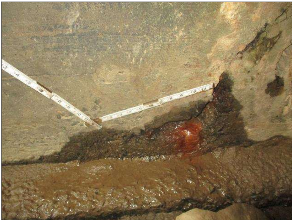
Span 1 Culvert Section 1: 8 INCHES LONG X 3 INCHES HIGH X 4 INCHES DEEP SPALLED AREA IN THE WEST WALL, 3 FEET FROM THE DOWNSTREAM END OF THE BARREL
