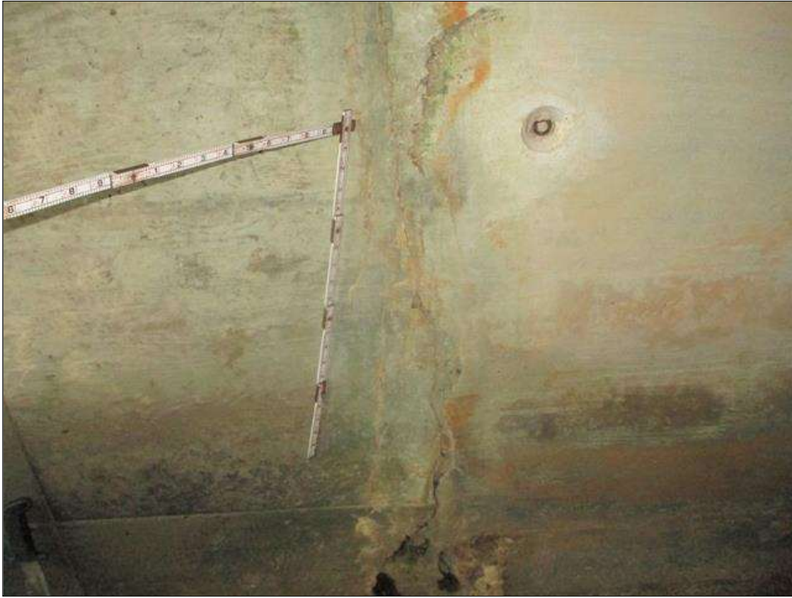
Span 1 Culvert Section 1: FULL HEIGHT X FULL WIDTH X UP TO 1/4 INCHES WIDE VERTICAL WRAP AROUND CRACK WITH EFFLORESCENCE AND SPALLED AND DELAMINATED AREAS UP TO 3 INCHES LONG X 4 INCHES HIGH X 1.5 INCHES DEEP IN THE WALLS AND TOP SLAB, 9.5 FEET FROM THE DOWNSTREAM END OF THE BARREL
