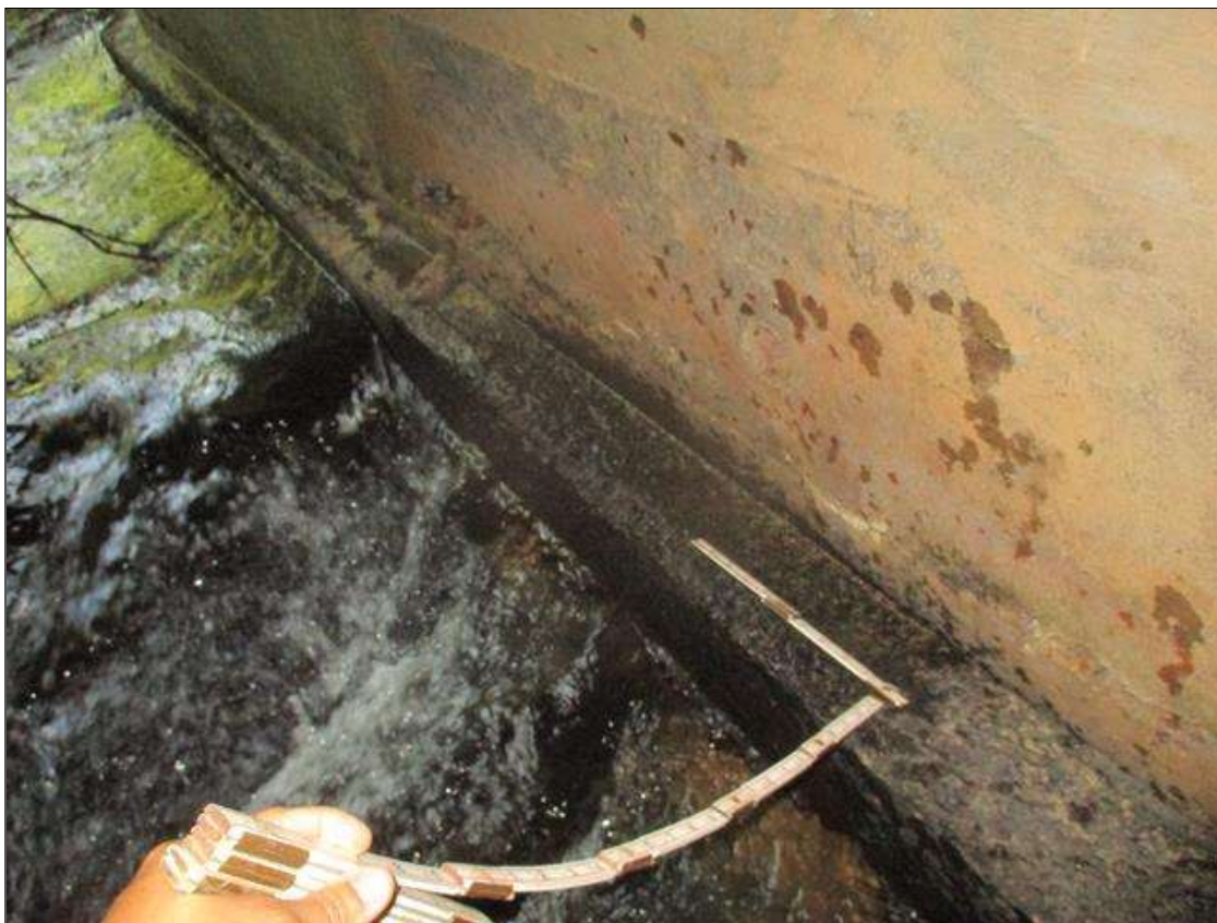
Span 3 Culvert Section 1: FULL LENGTH X FULL WIDTH X FULL HEIGHT SCALING THROUGHOUT THE EAST AND WEST FOOTINGS
