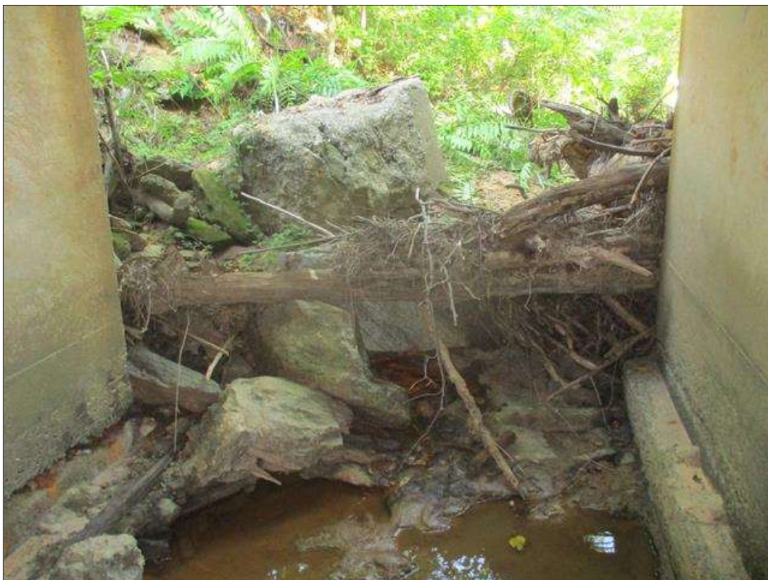
Span 1 Culvert Section 1: UP TO 3 FEET X 1 FEET X 2 INCHES SCOUR AT UPSTREAM END OF BARREL 1 (SCOUR WAS COVERED BY DRIFT DURING 2023 INSPECTION)
