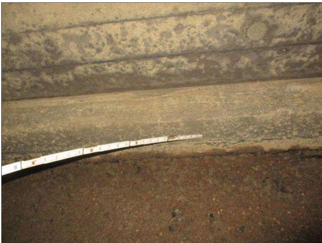
Span 2 Culvert Section 1: FULL LENGTH X FULL WIDTH X FULL HEIGHT SCALING THROUGHOUT THE EAST AND WEST FOOTINGS.
