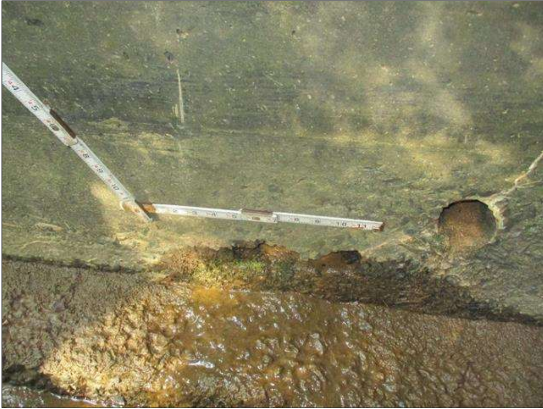
Span 1 Culvert Section 1: 8 INCHES LONG X 10 INCHES HIGH X UP TO 2 INCHES SPALLED AREA IN THE WEST WALL AT THE FOOTING, 9 FEET FROM THE DOWNSTREAM END OF THE BARREL
