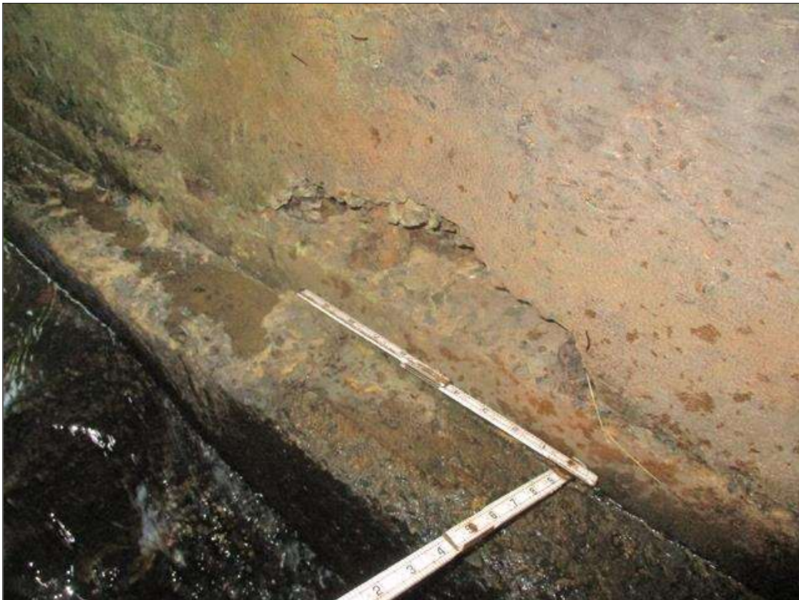
Span 3 Culvert Section 1: INTERMITTENT 14.5 FEET LONG X 7 INCHES HIGH X 5 INCHES DEEP SPALLED AREA 4 INCHES ABOVE THE FOOTING AT THE UPSTREAM END
