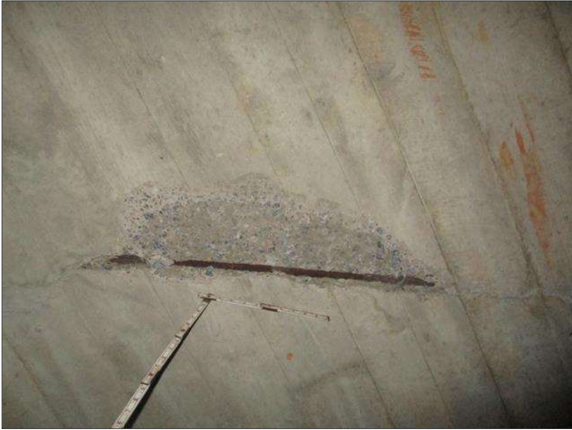
Span 1 Culvert Section 1: INTERMITTENT FULL WIDTH X 1.167 FEET LONG X 1.5 INCHES DEEP SPALLED AND DELAMINATED AREA WITH EXPOSED REINFORCEMENT IN THE TOP SLAB, 45 FEET FROM THE UPSTREAM END OF THE BARREL
