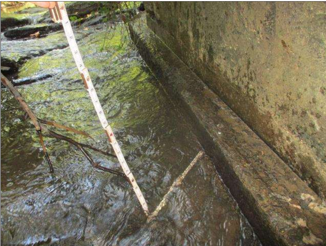
Span 3 Culvert Section 1: (PAR) 5 FEET LONG X 8 INCHES HIGH X 8 INCHES DEEP UNDERMINING OF THE EAST FOOTING, 4 FEET FROM THE UPSTREAM END OF THE BARREL
