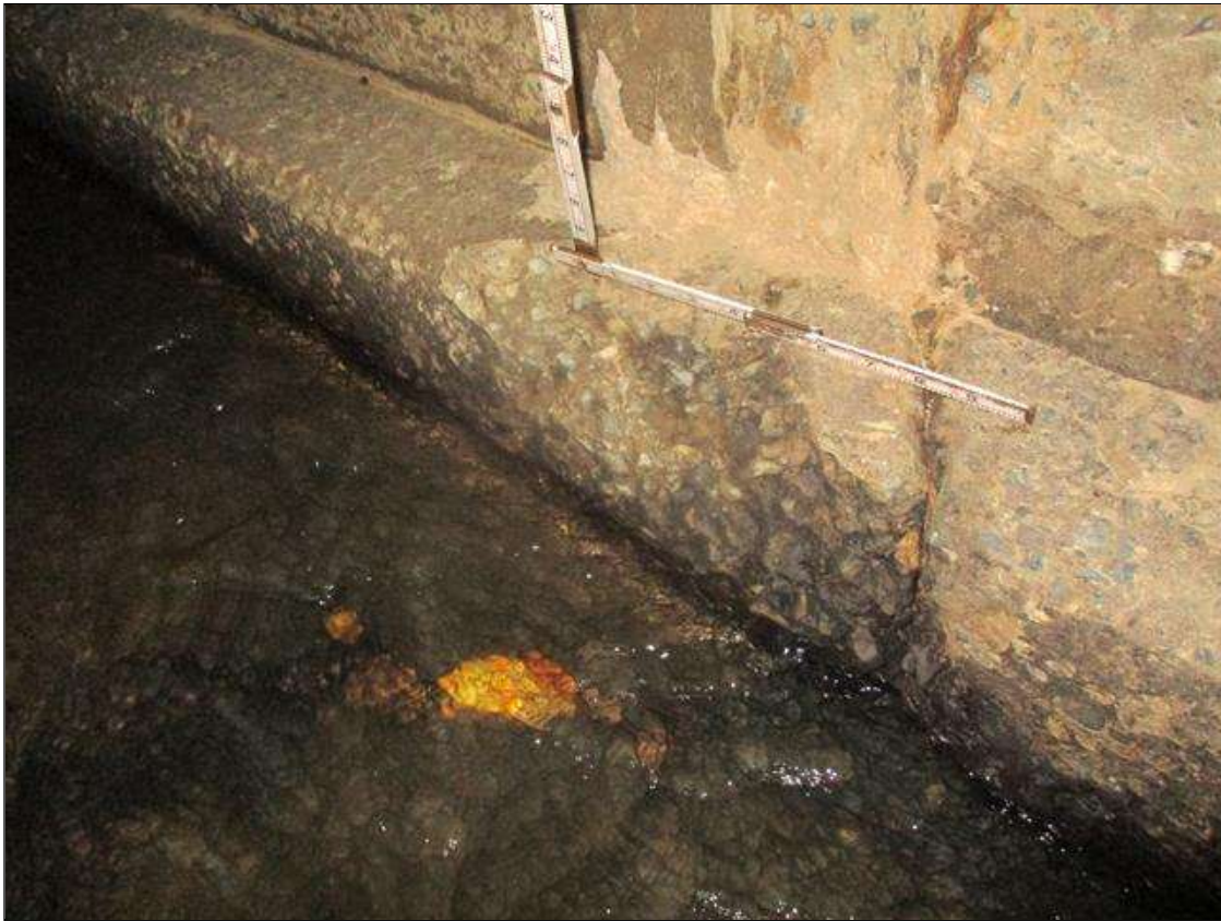
Span 3 Culvert Section 1: (8) UP TO 6 FEET X 5 INCHES X 5 INCHES SPALLS AT RANDOM THROUGHOUT EAST AND WEST FOOTINGS.
