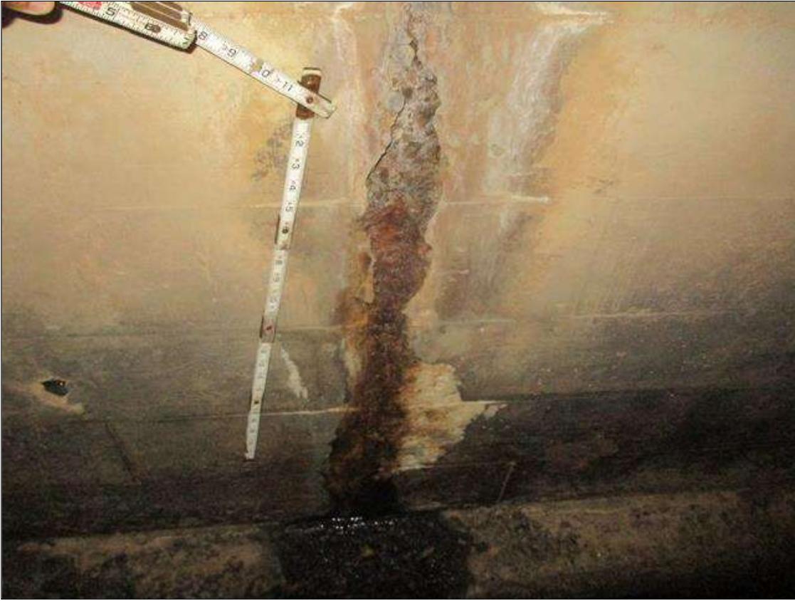
Span 3 Culvert Section 1: 1.25 FEET HIGH 3 INCHES LONG X 3/4 INCHES DEEP SPALLED AREA WITH A 6 FEET HIGH X 1/4 INCHES WIDE VERTICAL CRACK WITH EFFLORESCENCE AND HEAVY BUILDUP AND RUST STAINING ADJACENT TO 15 INCHES X 5 INCHES X 4 INCHES SPALL IN EAST FOOTING, 19 FEET FROM THE DOWNSTREAM END OF THE BARREL
