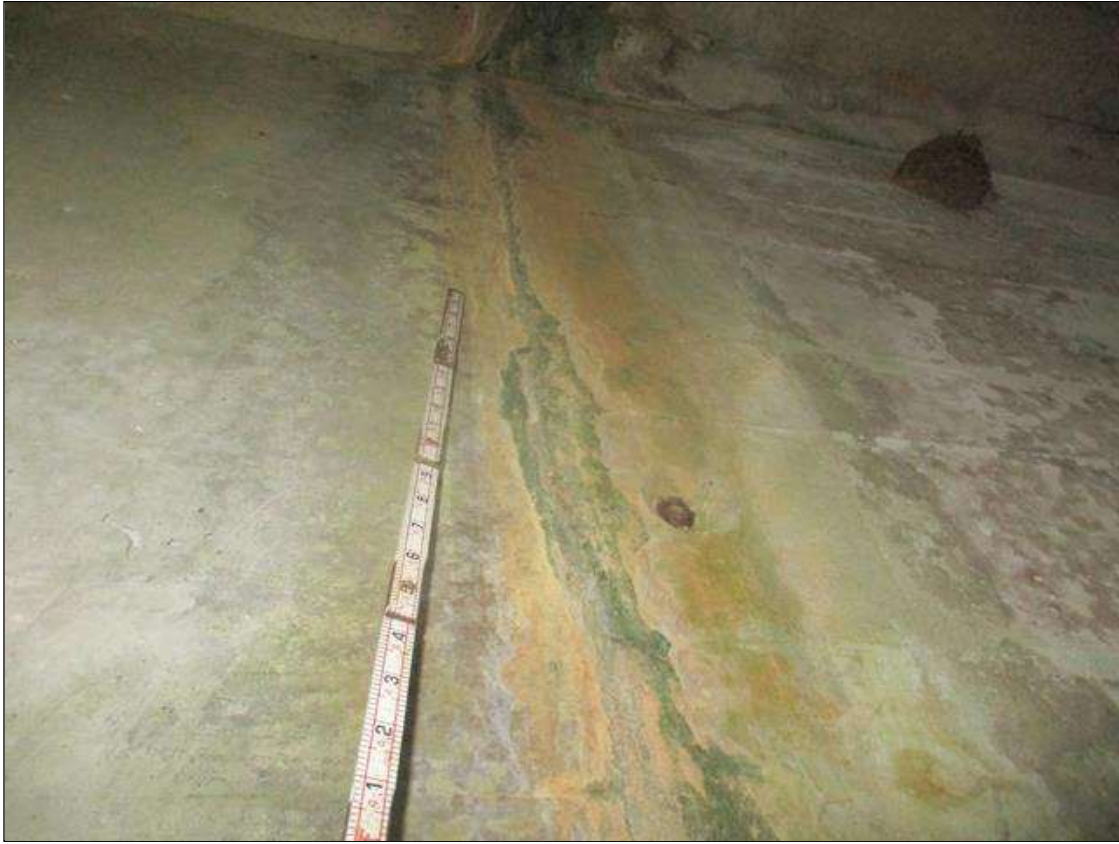
Span 2 Culvert Section 1: FULL HEIGHT X FULL WIDTH X UP TO 1/4 INCHES WIDE VERTICAL WRAP AROUND CRACK IN THE WALLS AND TOP SLAB WITH EFFLORESCENCE AND INTERMITTENT FULL WIDTH X 5 INCHES LONG DELAMINATION IN THE TOP SLAB AND UP TO 12 INCHES X 4 INCHES X 4 INCHES INTERMITTENT SPALLS, 9 FEET FROM THE DOWNSTREAM END OF THE BARREL
