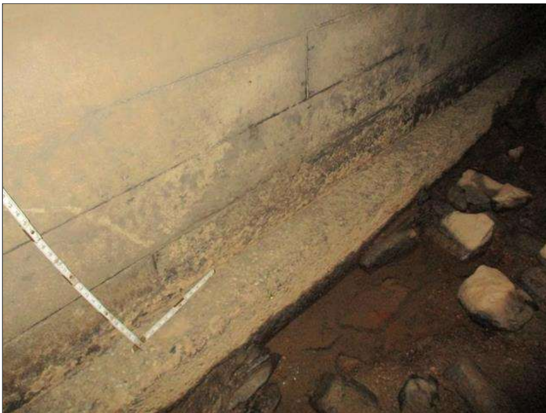
Span 1 Culvert Section 1: FULL LENGTH X FULL WIDTH X FULL HEIGHT SCALING THROUGHOUT THE EAST AND WEST FOOTINGS
