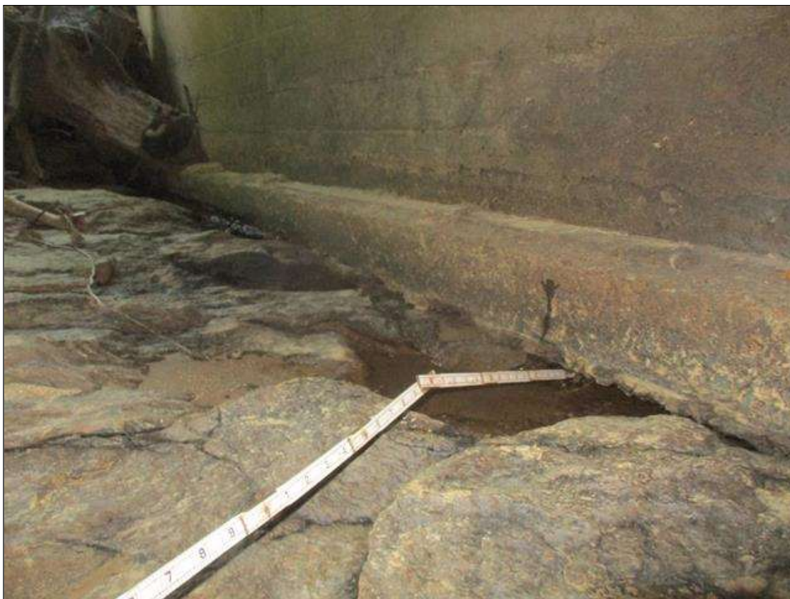
Span 2 Culvert Section 1: (PAR) 8 FEET LONG X 4 INCHES HIGH X FULL DEPTH UNDERMINING WITH WATER FLOW BENEATH THE EAST FOOTING BETWEEN BARREL 2 AND BARREL 3, 10 FEET FROM THE UPSTREAM END OF THE BARREL
