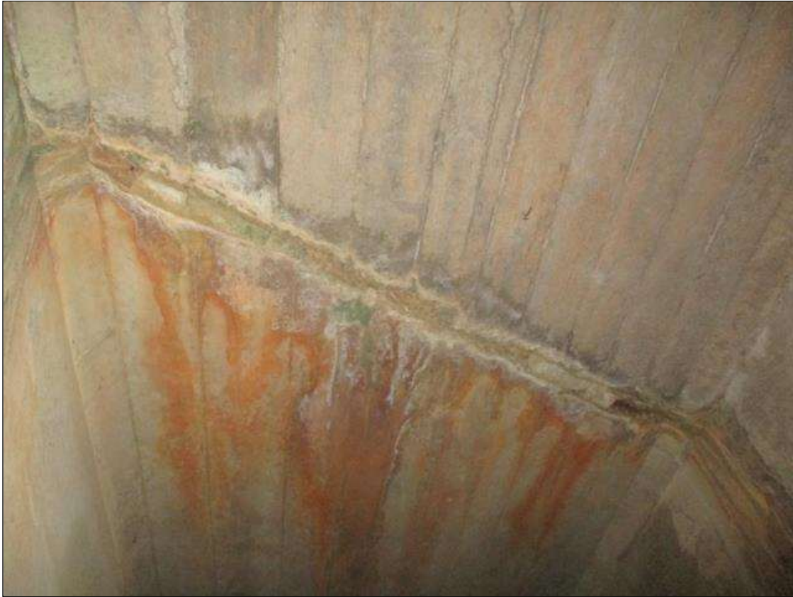
Span 2 Culvert Section 1: FULL HEIGHT X FULL WIDTH X UP TO 1/8 INCHES WIDE VERTICAL WRAP AROUND CRACK IN THE WALLS AND TOP SLAB WITH EFFLORESCENCE AND INTERMITTENT SPALLED AND DELAMINATED AREAS UP TO 12 INCHES X 18 INCHES X 4 INCHES IN THE WALLS AND TOP SLAB, 13.75 FEET FROM THE UPSTREAM END OF THE BARREL
