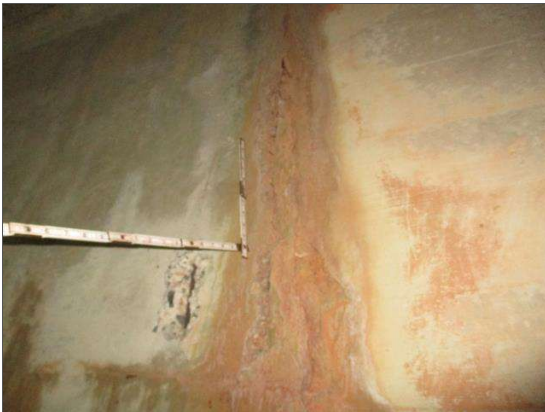
Span 3 Culvert Section 1: INTERMITTENT FULL HEIGHT X 1 FEET LONG X 1.5 INCHES DEEP SPALLED AND DELAMINATED AREA WITH A FULL HEIGHT X 1/8 INCHES WIDE VERTICAL CRACK IN THE EAST WALL, 14.5 FEET FROM THE UPSTREAM END OF THE BARREL
