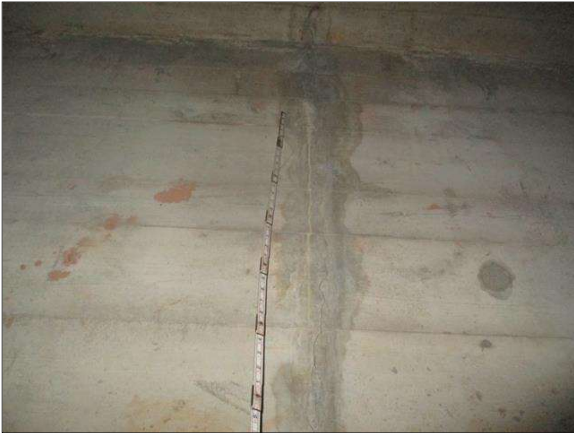
Span 2 Culvert Section 1: FULL HEIGHT X FULL WIDTH X UP TO 1/8 INCHES WIDE VERTICAL WRAP AROUND CRACKS WITH EFFLORESCENCE IN THE WALLS AND TOP SLAB AT GREATER THAN 3 FEET SPACING ALONG THE FULL LENGTH OF THE BARREL
