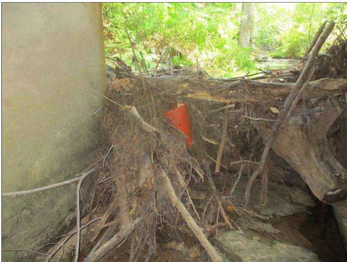
Span 2 Culvert Section 1: INTERIOR WALL 1 AT INLET, SPALL (15 INCHES X 7 INCHES X UP TO 3/4 INCH) (SCOUR WAS COVERED BY DRIFT DURING 2023 INSPECTION)
