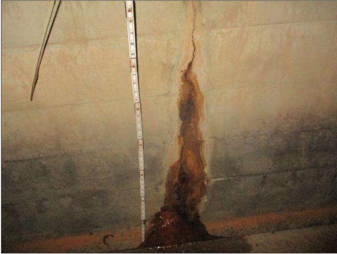
Span 1 Culvert Section 1: FULL HEIGHT X FULL WIDTH X UP TO 1/8 INCHES WIDE VERTICAL WRAP AROUND CRACKS WITH EFFLORESCENCE IN THE WALLS AND TOP SLAB AT GREATER THAN 3 FEET SPACING ALONG THE FULL LENGTH OF THE BARREL
