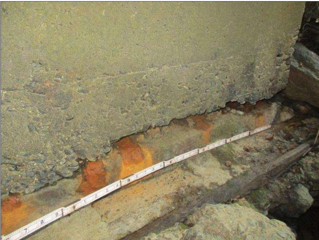
Span 1 Culvert Section 1: INTERMITTENT 14 FEET LONG X INTERMITTENT 10 INCHES HIGH X 3 INCHES DEEP SPALLED AREA IN THE WEST WALL AT THE FOOTING, AT THE UPSTREAM END OF THE BARREL
