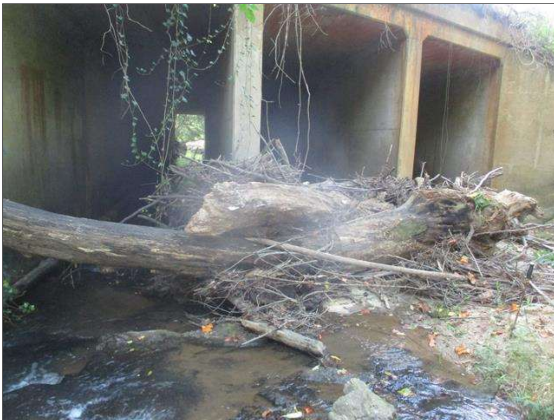
LARGE DRIFT ACCUMULATION AT INLET IN FRONT OF BARRELS 1 THROUGH 3
