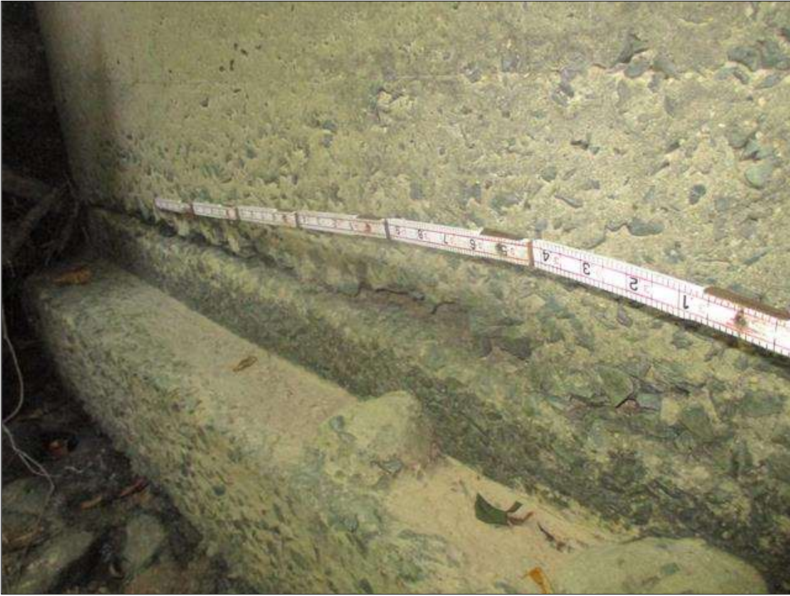
Span 1 Culvert Section 1: 4 FEET LONG X 4 INCHES HIGH X 2 INCHES DEEP SPALLED AREA IN THE EAST WALL AT THE FOOTING, AT THE UPSTREAM END OF THE BARREL
