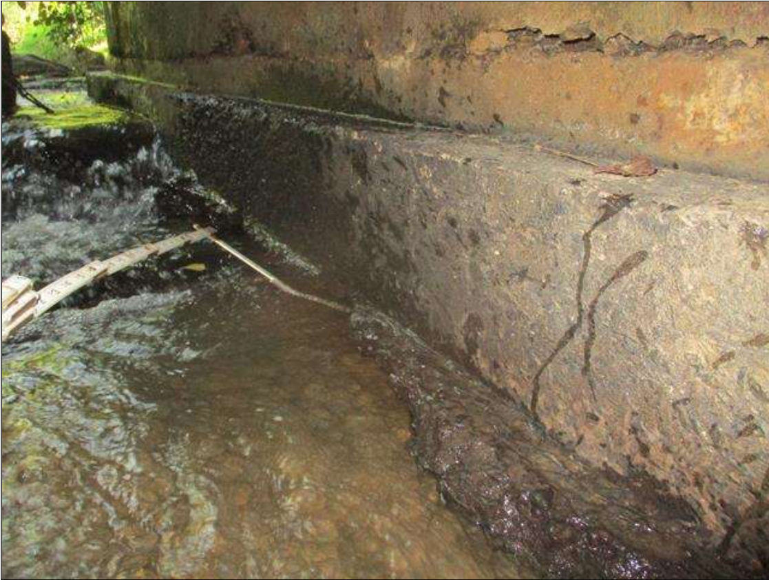
Span 3 Culvert Section 1: (PAR) 5 FEET LONG X 5 INCHES HIGH X 9 INCHES DEEP UNDERMINING OF THE EAST FOOTING, 9.5 FEET FROM THE UPSTREAM END OF THE BARREL
