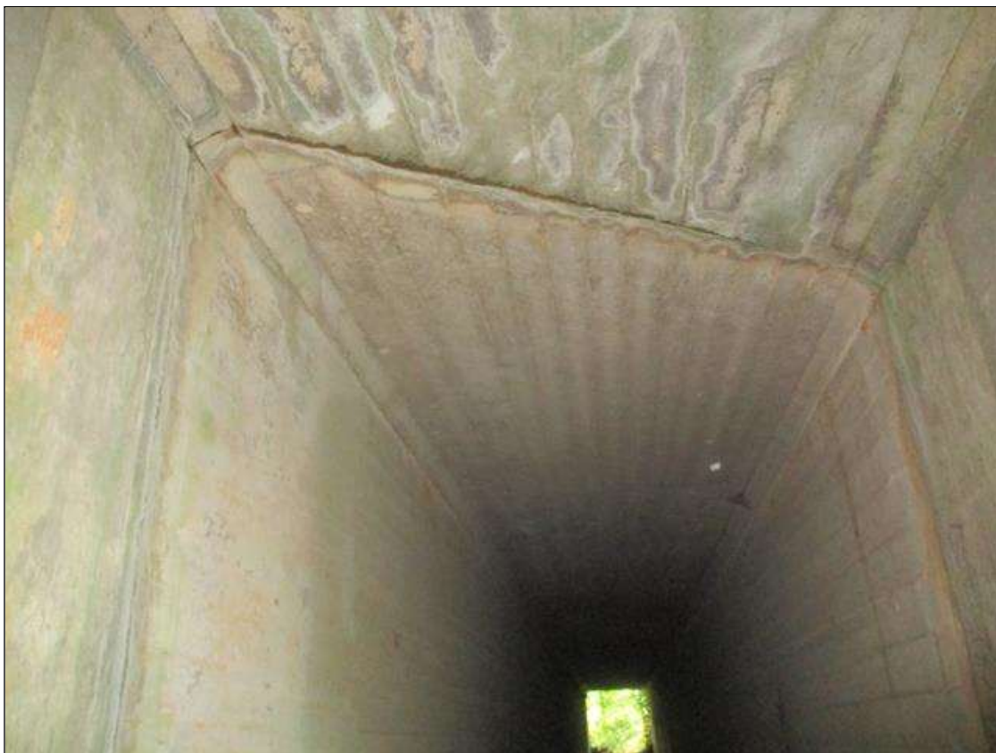
Span 3 Culvert Section 1: FULL HEIGHT X FULL WIDTH X UP TO 1/8 INCHES WIDE VERTICAL WRAP AROUND CRACKS WITH EFFLORESCENCE IN THE WALLS AND TOP SLAB AT GREATER THAN 3 FEET SPACING ALONG THE FULL LENGTH OF THE BARREL
