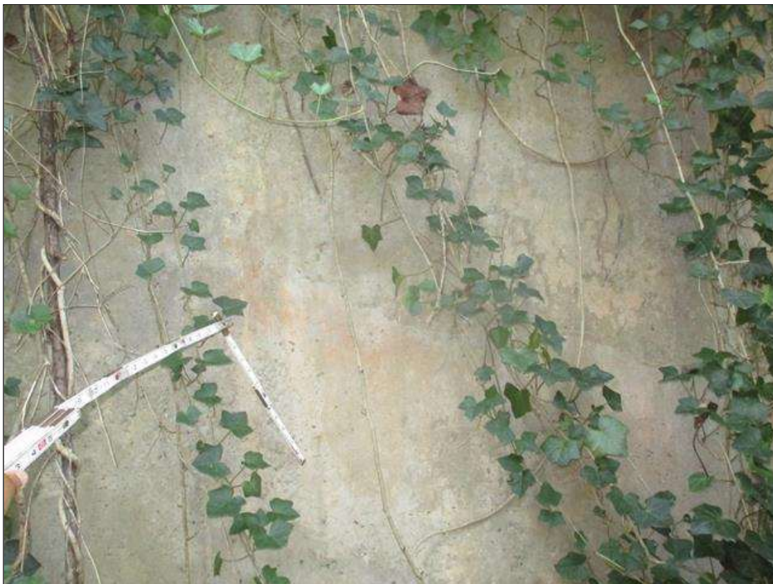
14 FEET X 10 FEET X UP TO 1/32 INCHES MAP CRACKING WITH RUST STAINING IN SOUTHWEST WINGWALL
