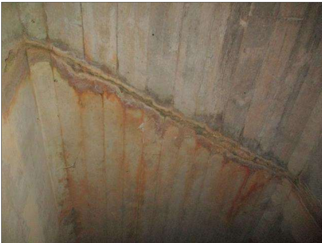
Span 3 Culvert Section 1: INTERMITTENT FULL WIDTH X 3 INCHES LONG DELAMINATED AREA WITH A FULL WIDTH X 1/4 INCHES WIDE TRANSVERSE CRACK IN THE TOP SLAB, 14.5 FEET FROM THE UPSTREAM END OF THE BARREL
