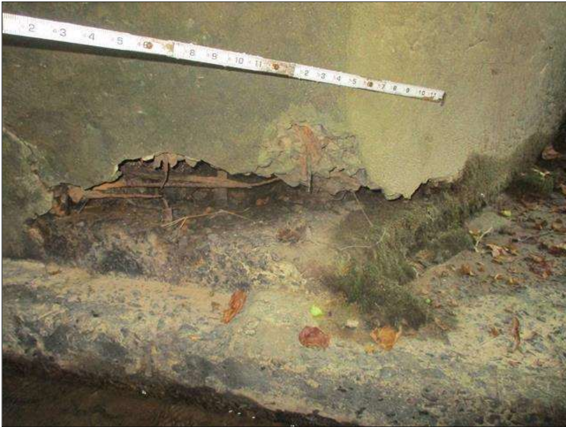
Span 3 Culvert Section 1: (PAR) 3 FEET LONG X 10 INCHES HIGH X 1 FOOT WIDE SPALLED AREA WITH EXPOSED AND BROKEN REINFORCEMENT, 1 FOOT DEEP UNDERMINING, AND EXPOSED FILL AT THE DOWNSTREAM END OF THE EAST WALL
