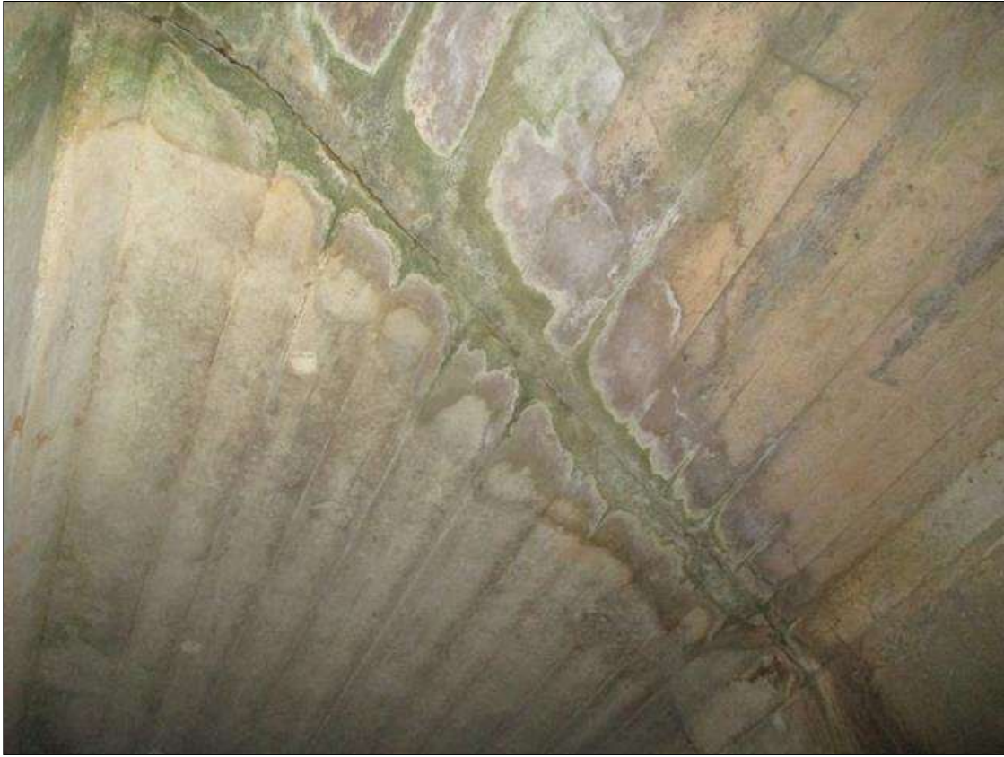
Span 1 Culvert Section 1: FULL HEIGHT X FULL WIDTH X UP TO 1/4 INCHES WIDE VERTICAL WRAP AROUND CRACK WITH EFFLORESCENCE AND SPALLED AND DELAMINATED AREAS UP TO 3 INCHES LONG X 4 INCHES HIGH X 1.5 INCHES DEEP IN THE WALLS AND TOP SLAB, 9.5 FEET FROM THE DOWNSTREAM END OF THE BARREL
