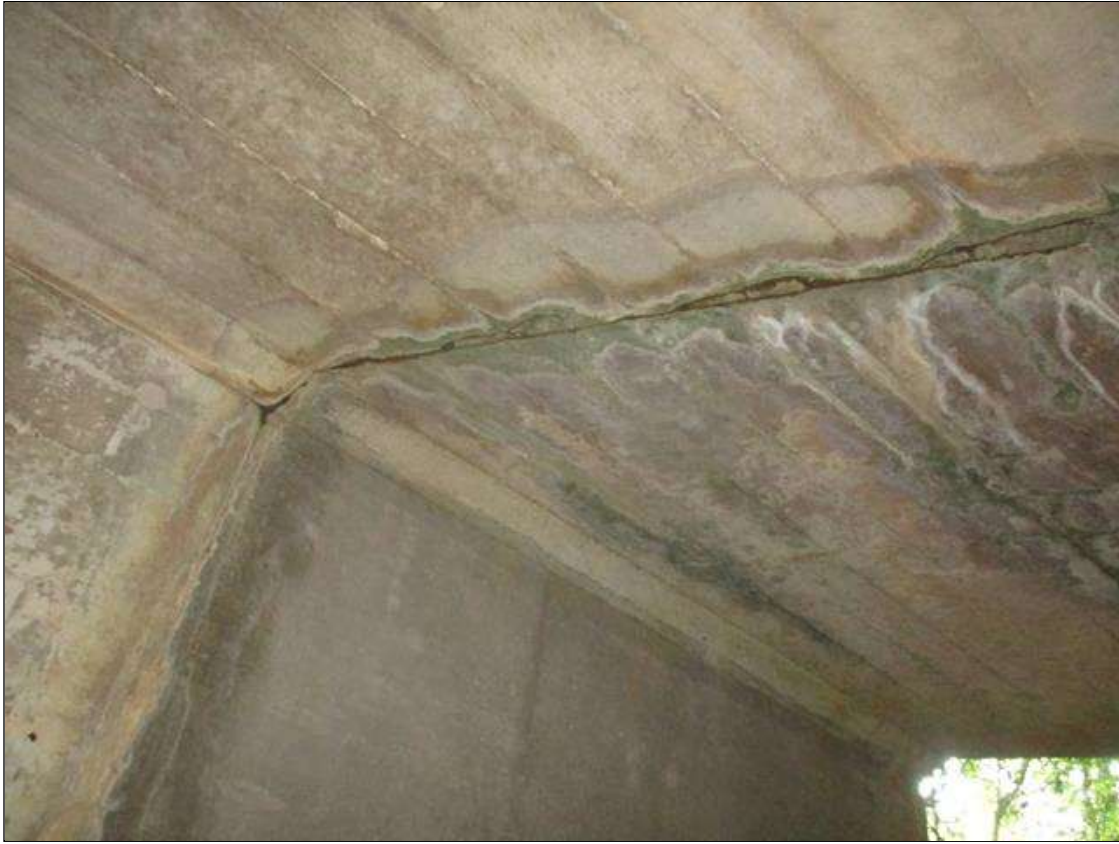
Span 2 Culvert Section 1: FULL HEIGHT X FULL WIDTH X UP TO 1/4 INCHES WIDE VERTICAL WRAP AROUND CRACK IN THE WALLS AND TOP SLAB WITH EFFLORESCENCE AND INTERMITTENT FULL WIDTH X 5 INCHES LONG DELAMINATION IN THE TOP SLAB AND UP TO 12 INCHES X 4 INCHES X 4 INCHES INTERMITTENT SPALLS, 9 FEET FROM THE DOWNSTREAM END OF THE BARREL
