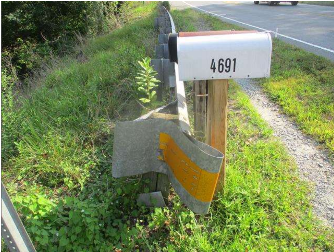
(PAR) IMPACT DAMAGE WITH SURFACE SCRAPES AT NORTHWEST GUARDRAIL TERMINAL END
