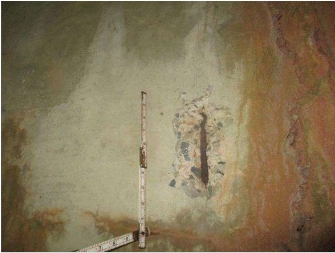
Span 3 Culvert Section 1: 8 INCHES HIGH X 4 INCHES LONG X 1 INCHES DEEP SPALLED AREA WITH EXPOSED REINFORCEMENT IN THE EAST WATERLINE, 4.5 FEET BELOW THE TOP SLAB, 13.5 FEET FROM THE UPSTREAM END OF THE BARREL
