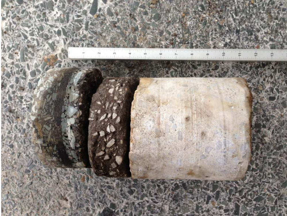
Exhibit A-22: Photograph of pavement core HA-05
