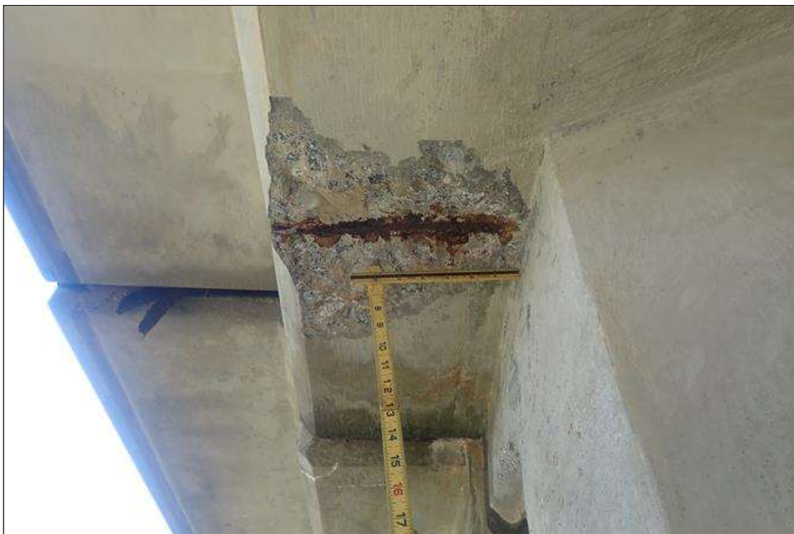
Span 2 Deck: (PAR) left overhang, at bent 2, spall (10 inch x 12 inch x 1.5 inch deep) with exposed rusted rebar
