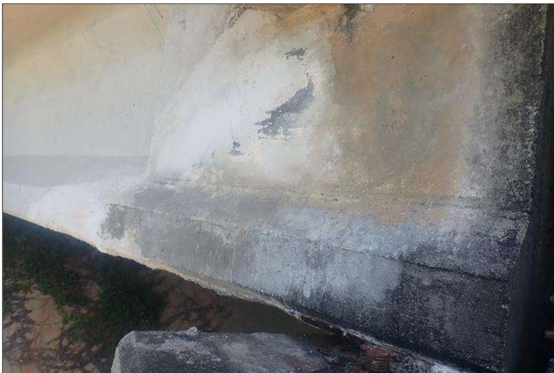
Span 4 Beam 1: 6 FOOT LONG X UP TO FULL HEIGHT PATCHED AREA THAT IS SOUND ON LEFT SIDE OF WEB AND BOTTOM FLANGE AT PIER 3.
