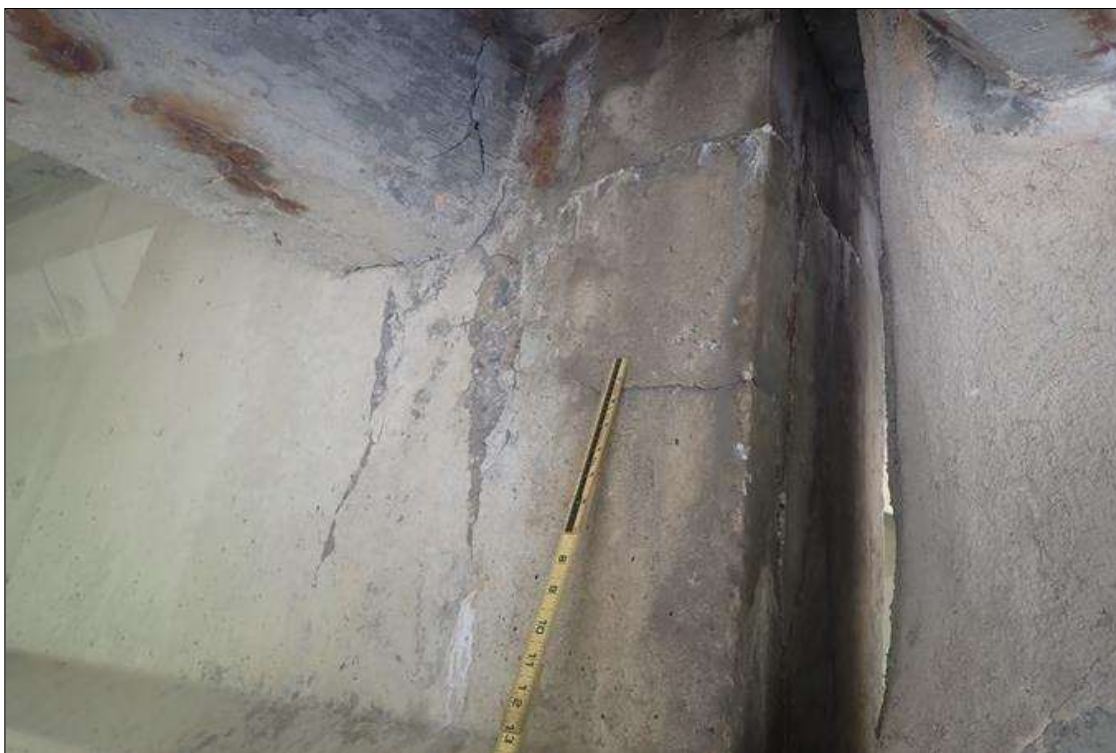
Span 1 Beam 2: (PAR) at bent 1, right face, delamination/spall (19 inches x full height x up to 3/4 inch deep) with efflorescence and rust stains
