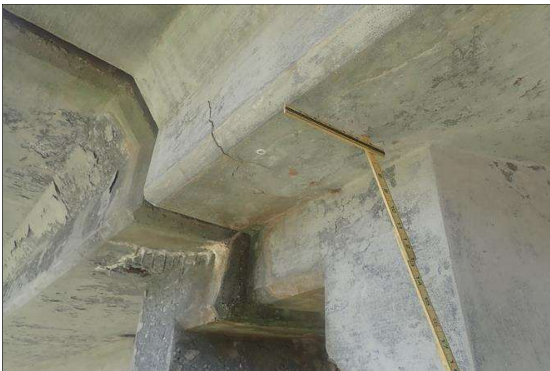
Span 3 Deck: right overhang, at bent 2, delamination (6 inch x 2 feet) with cracks (1/16 inch)
