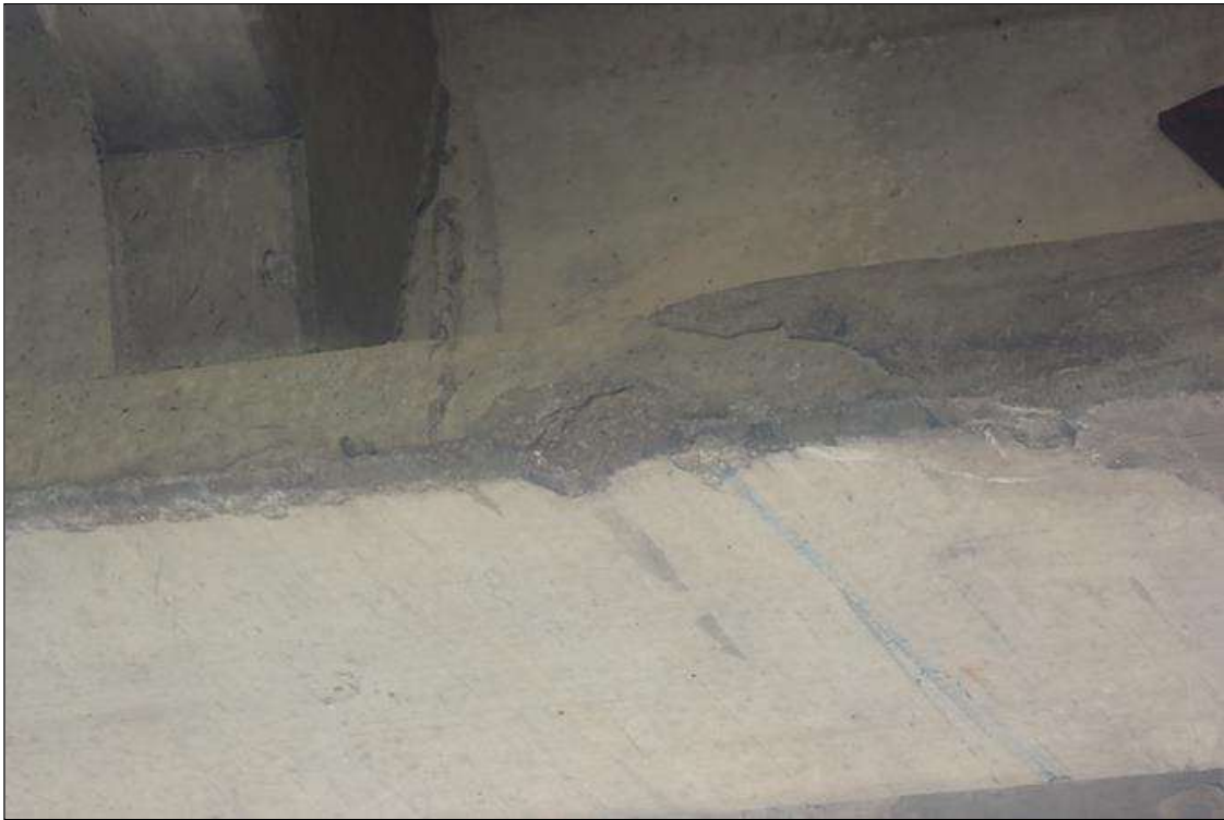
Span 3 Beam 2: (PAR) 07/07/2023 no apparent change since supplemental inspection, previously noted as: IMPACT DAMAGE - LOCATED 16 FEET FROM BENT 3; DIMENSIONS ARE 10 INCHES LONG X 5 INCHES HIGH X 1.25 INCHES DEEP
