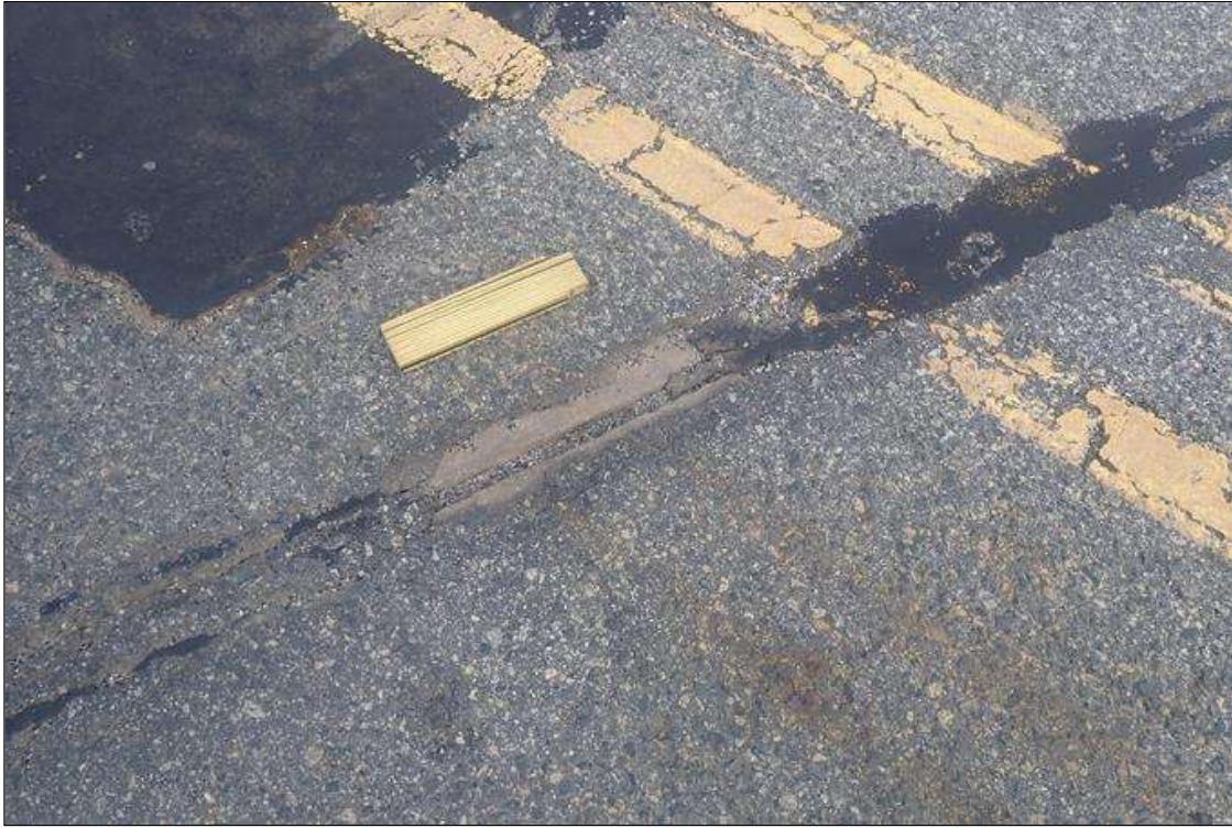
Span 2 Wearing Surface: 14 INCH LONG X 3 INCH WIDE X FULL DEPTH SPALL IN ASPHALT WEARING SURFACE EXPOSING JOINT OVER BENT 1
