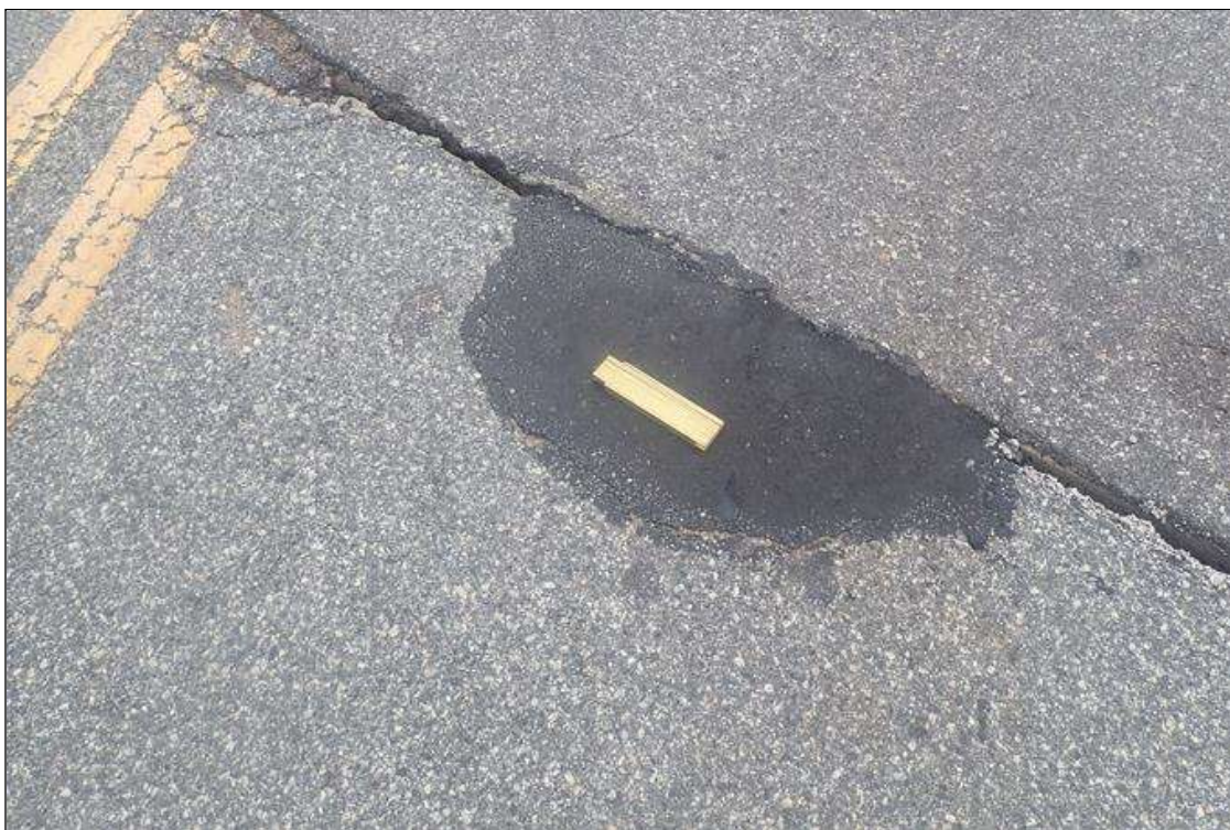
Span 4 Wearing Surface: southbound lane, at bent 3, patch (2.5 feet x 1.5 feet)
