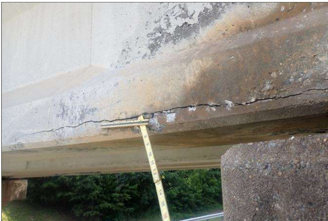
Span 3 Beam 1: (PAR) at bent 2, bottom flange, left face, longitudinal cracks (up to 1/8 inch x 4 feet)
