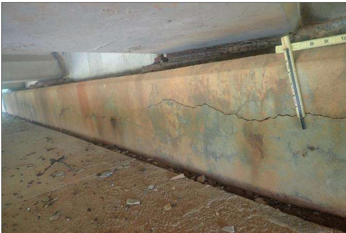
End Bent 1 Cap 1: (PAR) HORIZONTAL CRACK UP TO 3/16 INCH WITH DELAMINATION AND RUST STAINS ALONG FACE FOR FULL LENGTH
