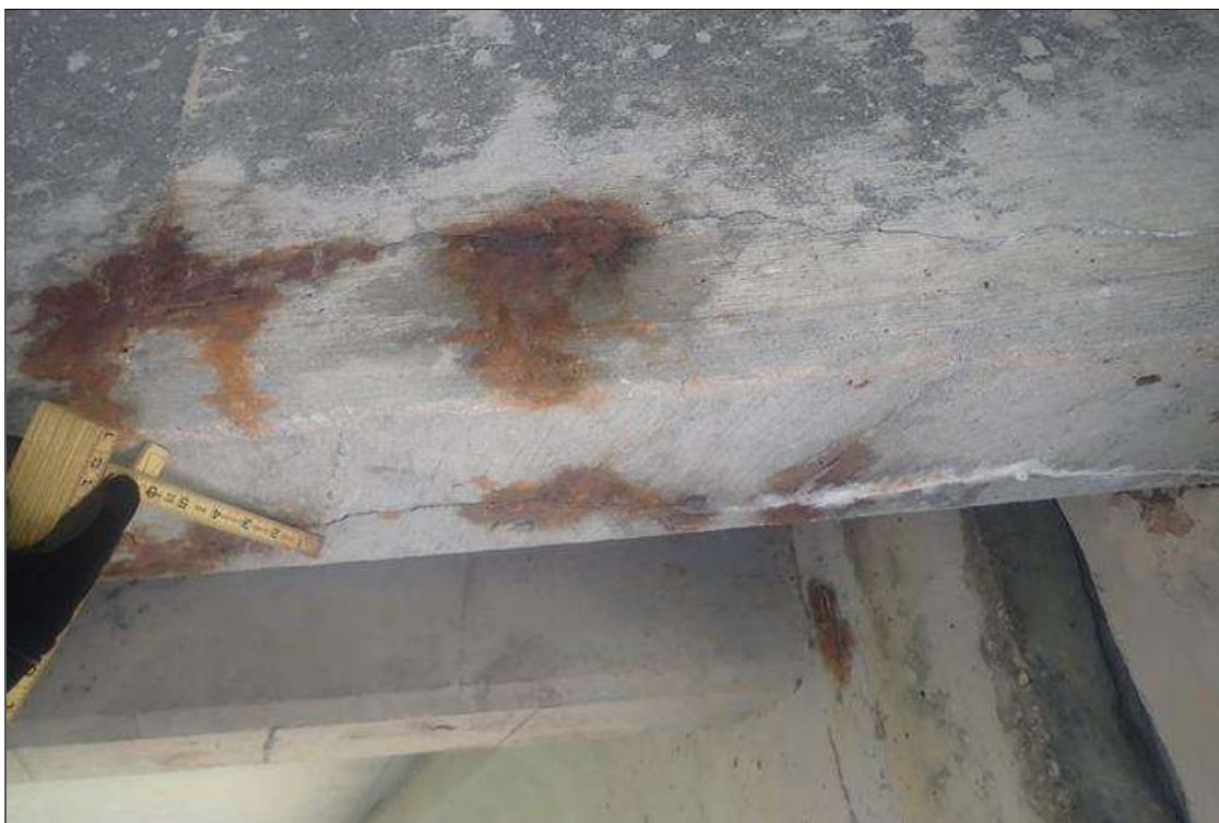
Span 2 Deck: (PAR) bent 1 end diaphragm, bays 1, 2, 3 and right overhang, longitudinal cracks (up to 1/8 inch x 6 feet long) with rust stains and some efflorescence buildup
