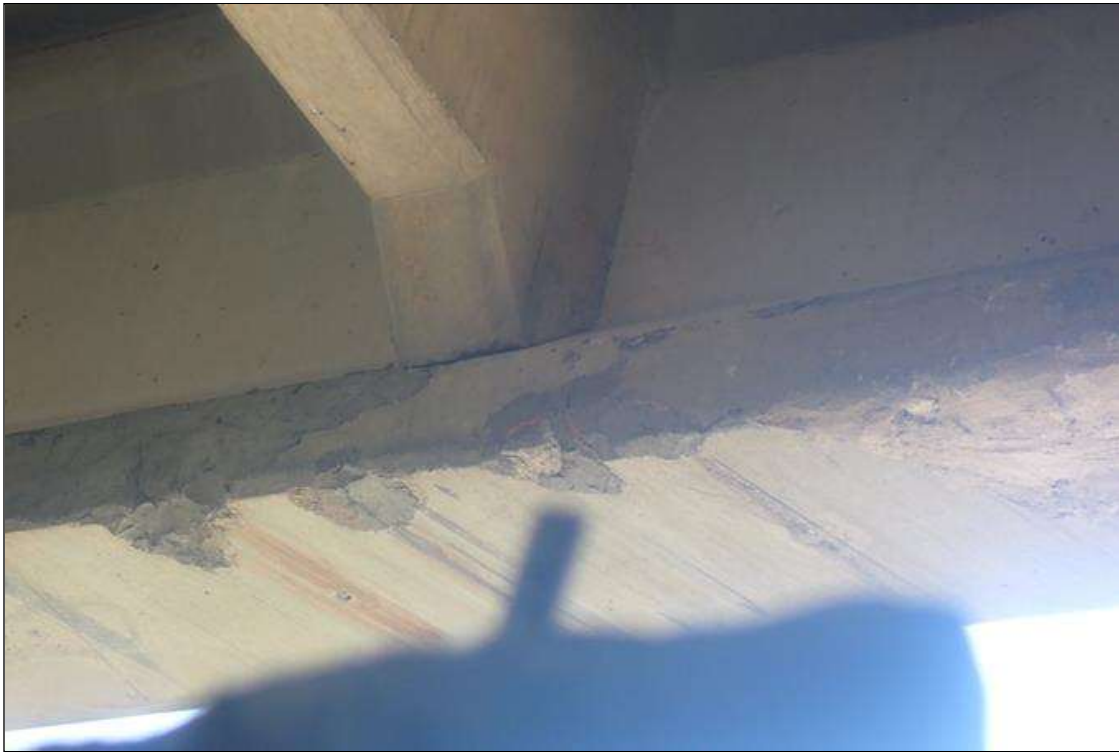
Span 3 Beam 1: (PAR) 07-07-2023 no change since supplemental inspection, right corner, previously noted as: IMPACT DAMAGE - LOCATED 19 FEET 4 INCHES FROM BENT 3; DIMENSIONS ARE 4 INCHES LONG X 3 INCHES HIGH X 1/2 INCH DEEP
