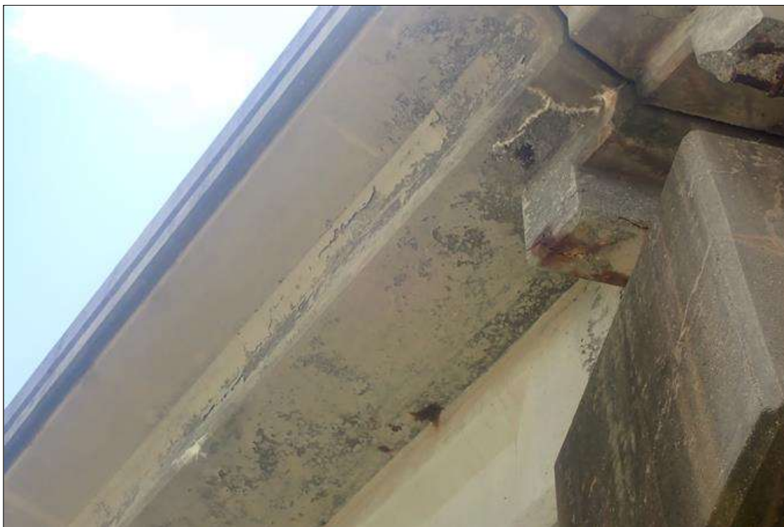
Span 2 Deck: (PAR) right overhang, near bent 2, (3) longitudinal/transverse cracks (hairline x 12 inch) with efflorescence buildup
