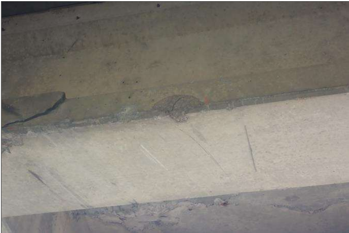
Span 3 Beam 2: (PAR) 07/07/2023 no apparent change since supplemental inspection, previously noted as: IMPACT DAMAGE- LOCATED 11 FEET 4 INCHES FROM BENT 3 WITH DIMENSIONS OF 1 FOOT 6 INCHES WIDE X 5 INCHES HIGH X 1/2 INCH DEEP
