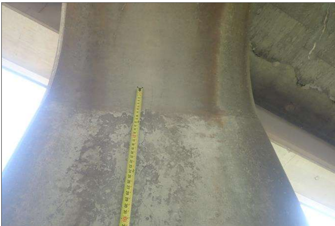
Bent 2 Pile 1: east face, at top, vertical crack (1/32 inch x 3 feet)
