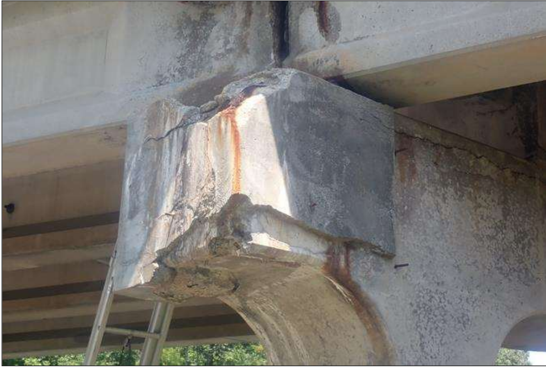
Bent 1 Cap 1: (PAR) west end of cap, delaminated/partially failed previous repair (3.5 feet long x full height x full width), with spalls (up to 2 feet x 16 inch x 2 inch deep) with exposed rusted rebar, rust stains, efflorescence buildup, and cracks (up to 1/8 inch)
