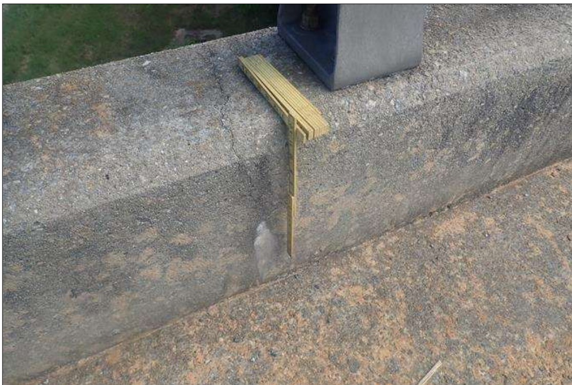
Span 1 Right Bridge Rail: parapet, at midspan, transverse crack (1/32 inch x full height) with efflorescence
