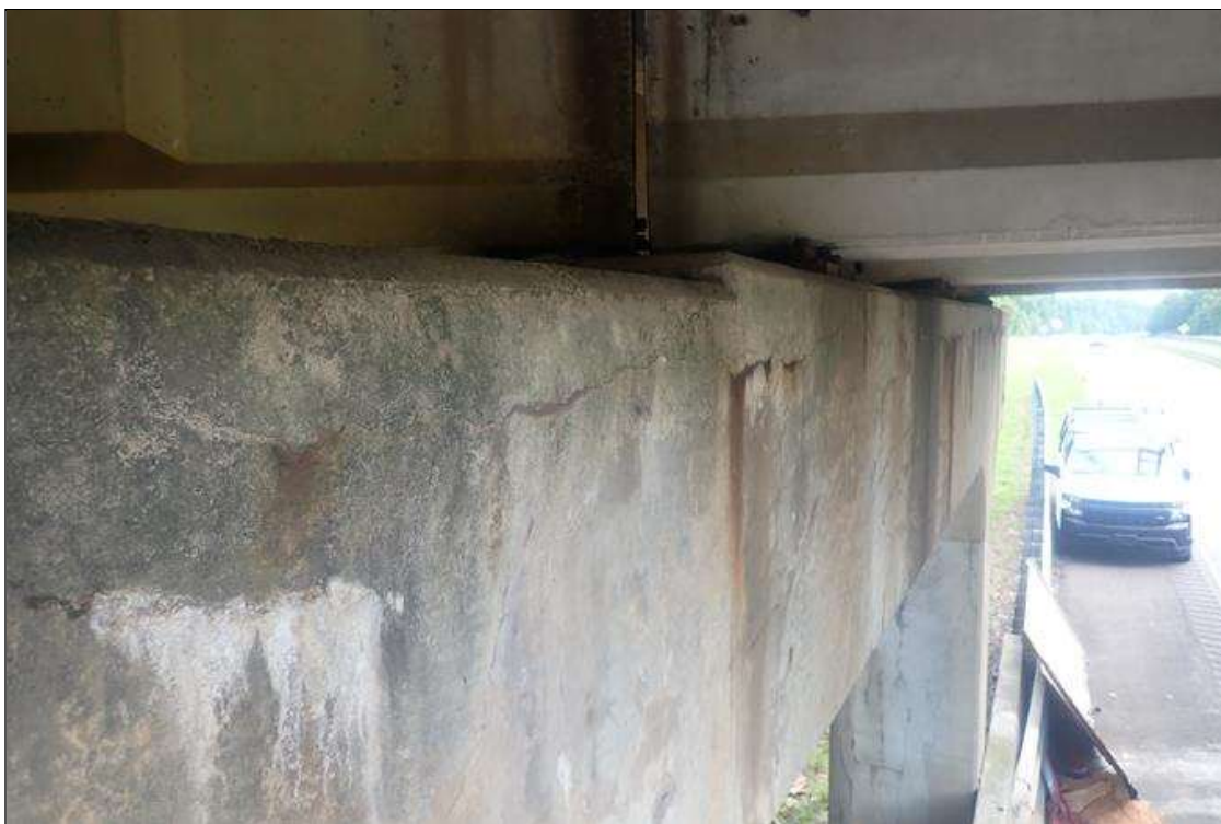
Bent 3 Cap 1: (PAR) 1/8 inch Horizontal crack on both faces of cap near top full length, with rust stains and some efflorescence buildup
