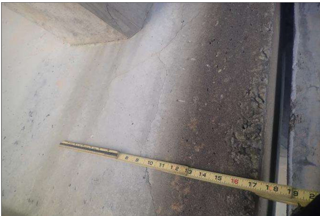
Span 4 Beam 2: (PAR) at bent 3, left face, web, map cracks (up to 0.018 inch x 16 inch x 30 inch)
