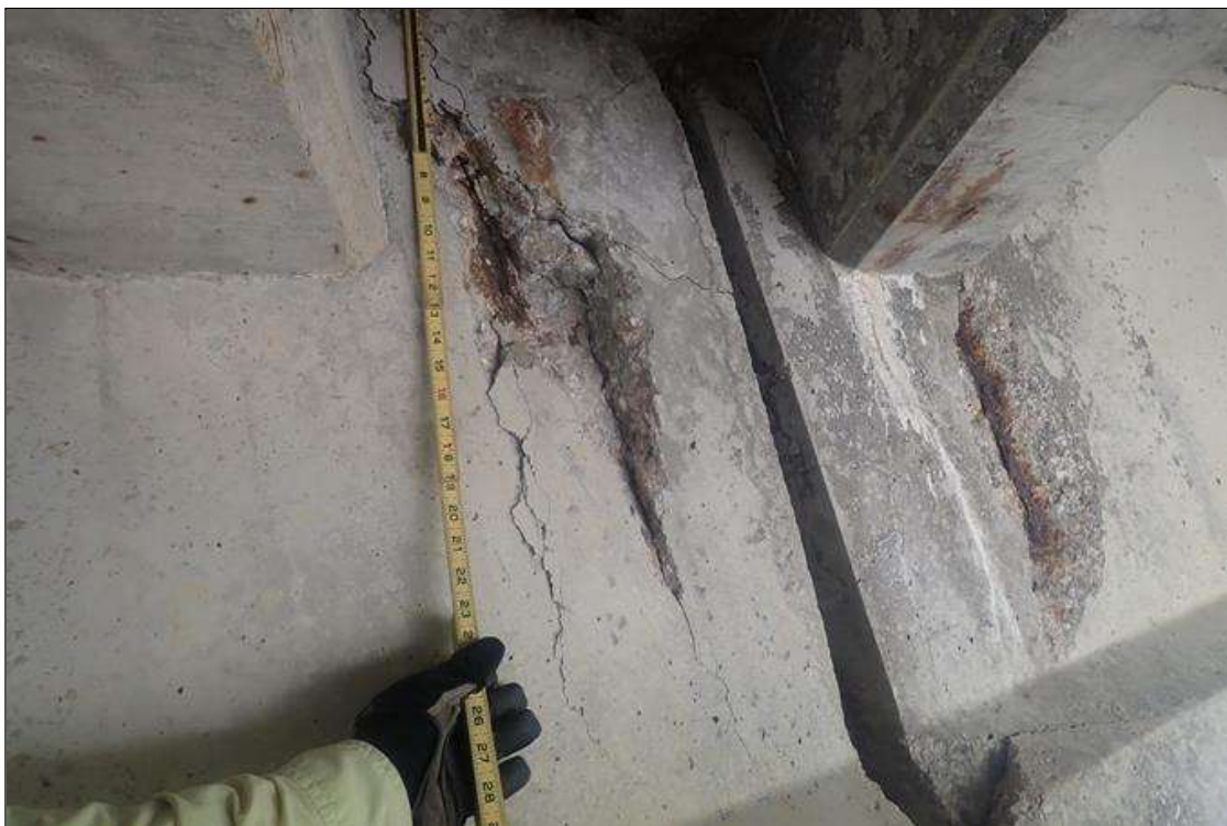
Span 3 Beam 3: 30 INCHES HIGH X 8 INCHES WIDE X 2 INCHES DEEP SPALL AND DELAMINATION ON LEFT SIDE WEB WITH EXPOSED STEEL OVER PIER 2. EXPOSED STEEL HAS NO MEASURABLE LOSS. SIMILAR RIGHT SIDE WEB.
