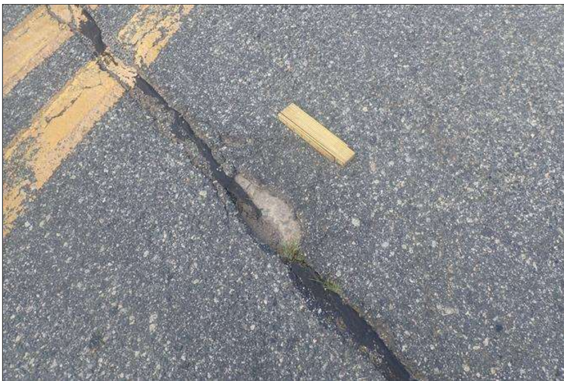
Span 1 Wearing Surface: 6 INCH LONG X 3 INCH WIDE X 1 INCH DEEP POTHOLE AT JOINT OVER END BENT 1
