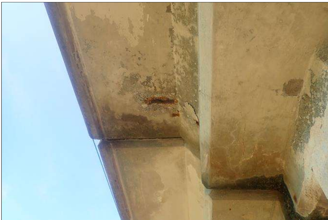
Span 3 Deck: (PAR) 6 INCH LONG X 4 INCHES WIDE X 3/4 INCH SPALL WITH EXPOSED RUSTED REBAR UNDER LEFT OVERHANG AT PIER 3
