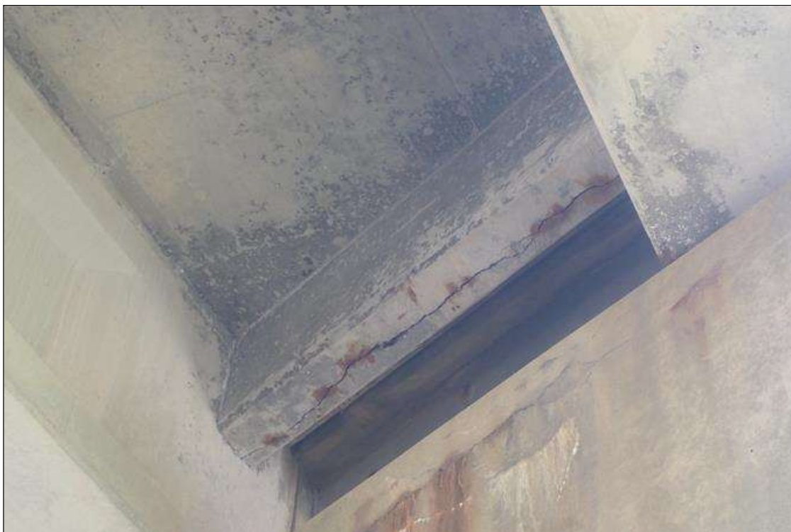
Span 2 Deck: (PAR) bent 2 end diaphragm, longitudinal crack (up to 1/4 inch x full length) with rust stains
