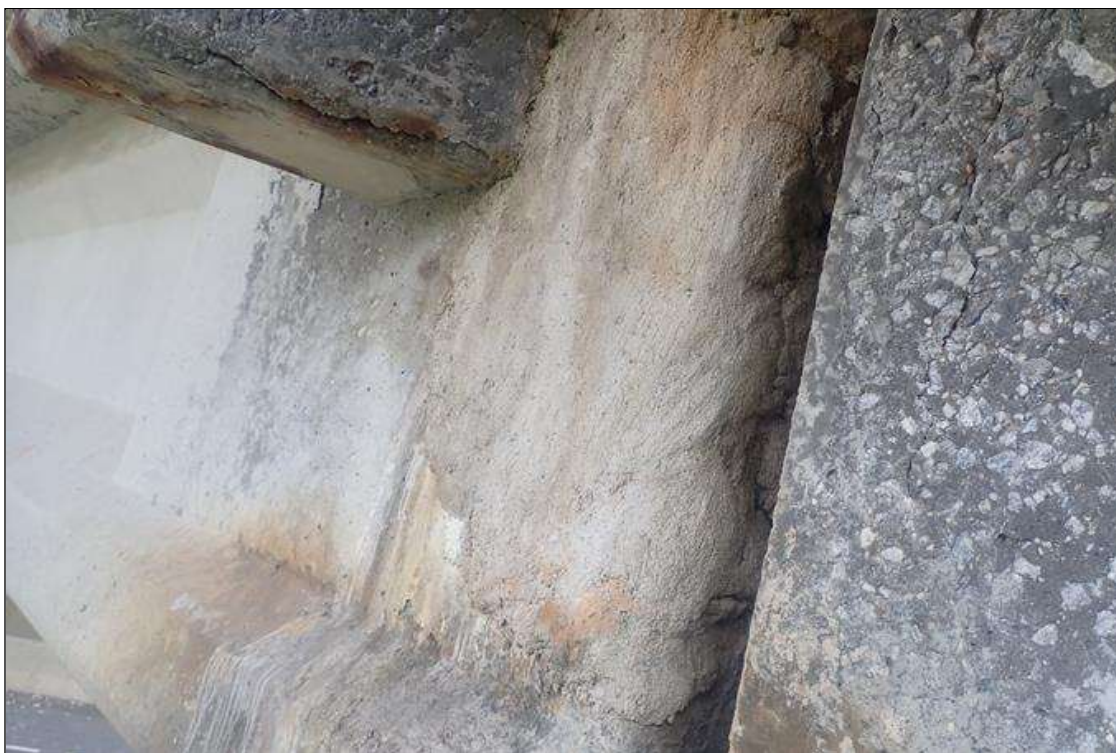
Span 2 Beam 4: Full height x 1 foot long sound patched area in right side of web at pier 2
