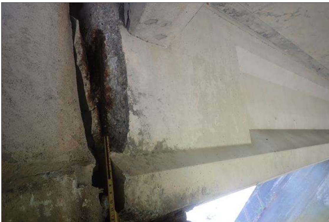
Span 1 Beam 3: (PAR) at bent 1, end of beam, both faces, spalls (up to 4 inch x 28 inch x 2.5 inch deep) with exposed rusted rebar
