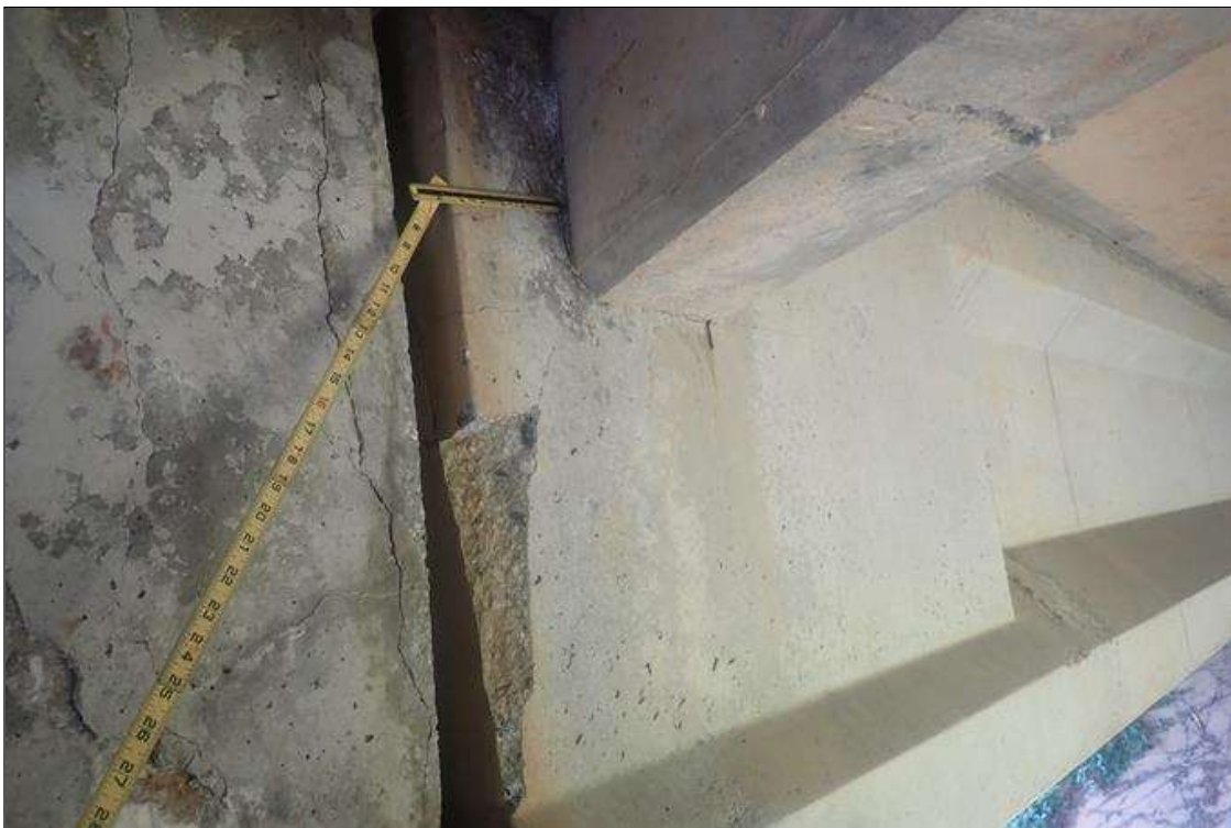
Span 4 Beam 3: at bent 3, end of web, spall/delamination (29 inch high x full width x up to 1.5 inch deep) with exposed rusted rebar extending along faces (up to 16 inches)
