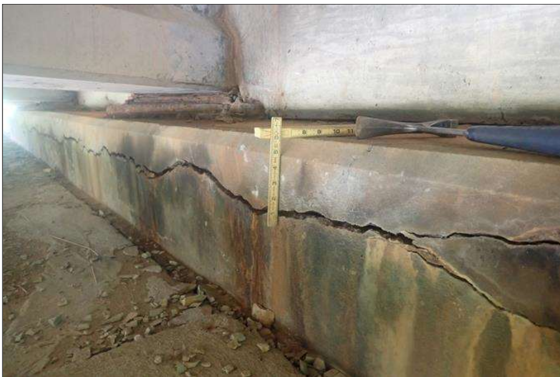
End Bent 2 Cap 1: (PAR) Full length area of delamination 12 inches high with horizontal cracks up to 3/4 inch with efflorescence and rust stains near top of cap which extend 6 inches on to top of cap.
