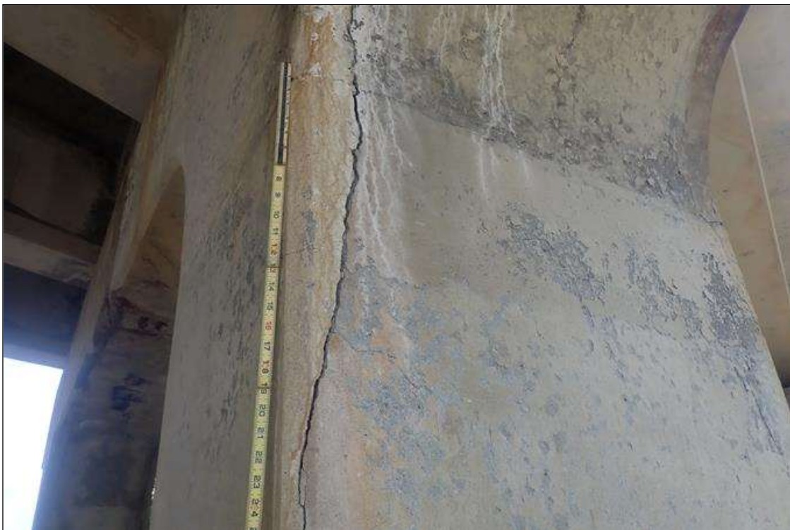
Bent 1 Pile 1: VERTICAL CRACKS UP TO 1/8 INCH ALONG EDGES FROM TOP DOWN 4 FEET WITH EFFLORESCENCE AND DELAMINATIONS (UP TO 6 INCH WIDE) AT WEST FACE CORNERS.
