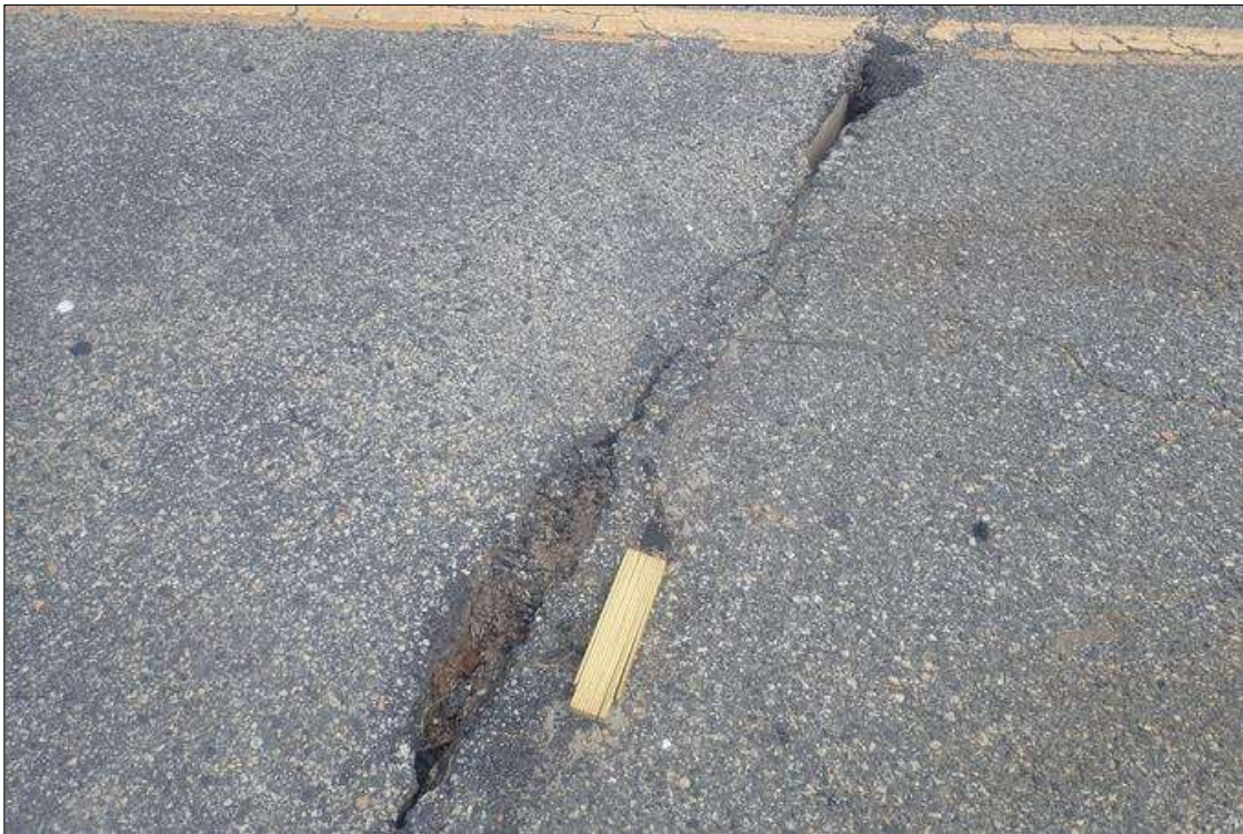
Span 3 Wearing Surface: southbound lane, over bent 2 joint, (2) potholes (up to 20 inch x 4 inch x full depth)
