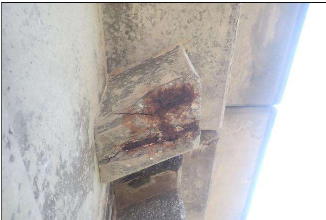
Span 2 Deck: bent 1 end diaphragm, left overhang, spall (16 inch x 8 inch x 2 inch deep) with exposed rusted rebar
