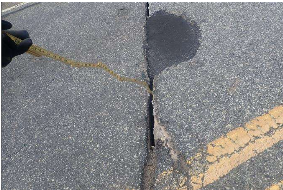
Span 4 Expansion Joint: southbound lane, joint material missing (9 feet)
