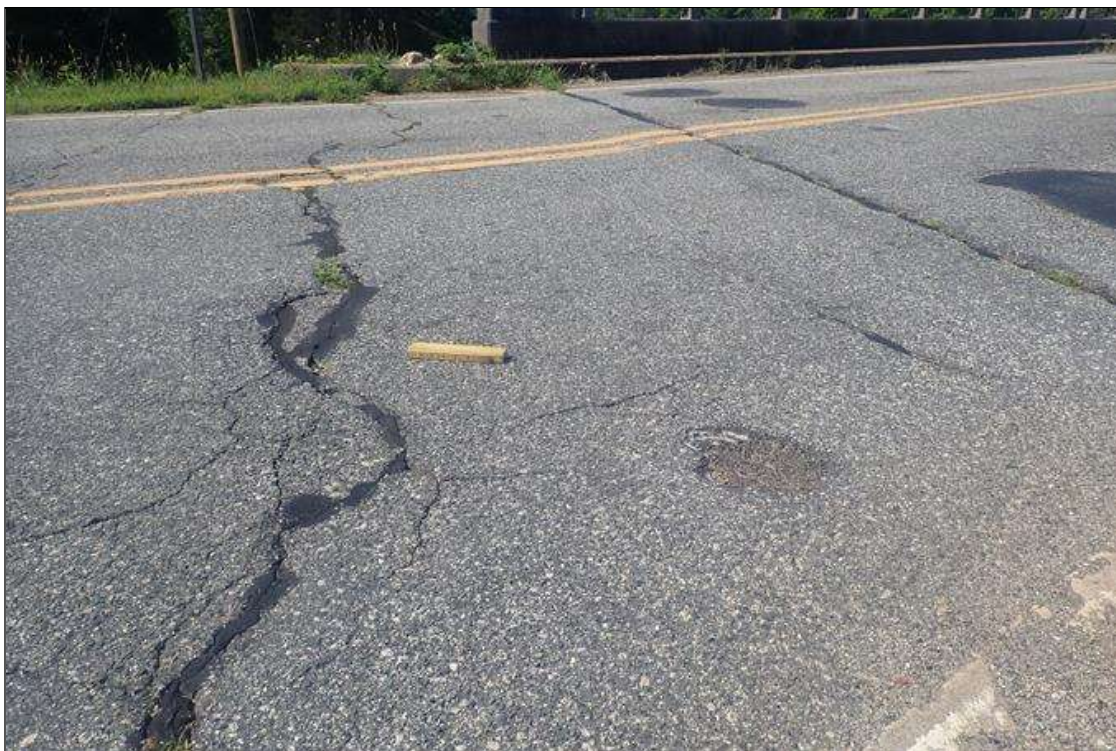
south approach asphalt, at bridge, transverse crack (up to 1/4 inch x full width) with settlement (7 feet x full width x approximately 1 inch deep)
