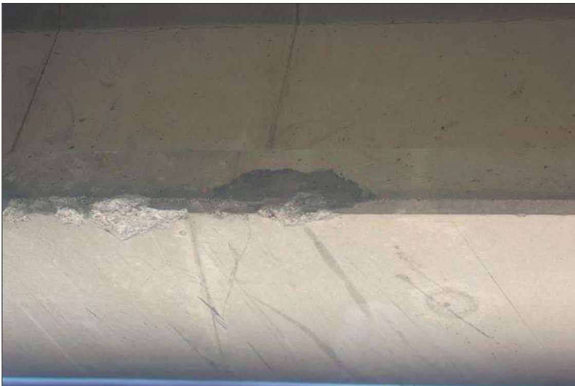
Span 3 Beam 1: (PAR) PATCHED AREAS THAT IS SOUND ALONG BOTTOM EDGE FROM IMPACT DAMAGE STARTING 12 FEET FROM PIER 3. - 02/16/2023 - IMPACT DAMAGE INSPECTION - LOCATED 12 FEET FROM BENT 3; DIMENSIONS ARE 7 INCHES LONG X 2 INCHES HIGH X 1 INCH DEEP ON PREVIOUS IMPACT REPAIR - 07-07-2023 no change since supplemental inspection, right corner
