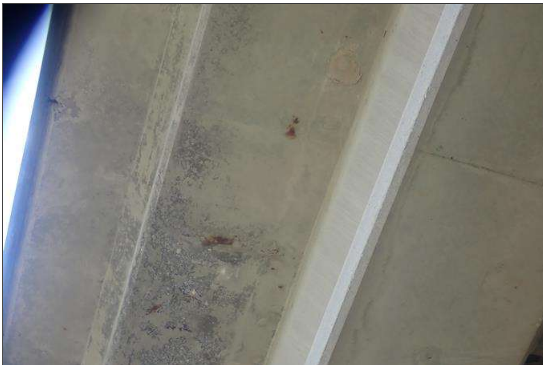
Span 3 Deck: (PAR) left overhang, at random, transverse cracks (hairline) with rust stains
