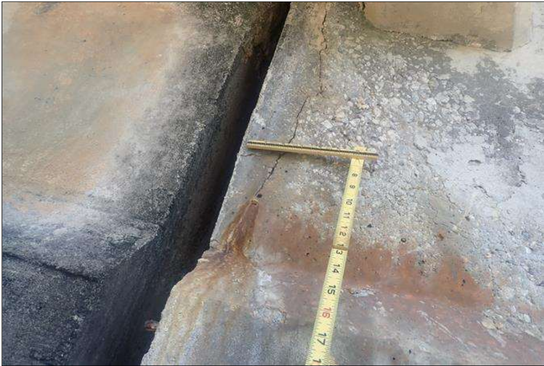
Span 3 Beam 1: (PAR) 1/16 INCH FULL HEIGHT VERTICAL CRACK, AND DELAMINATION (6 INCH WIDE), AND RUST STAINS IN LEFT SIDE OF WEB AT PIER 3.
