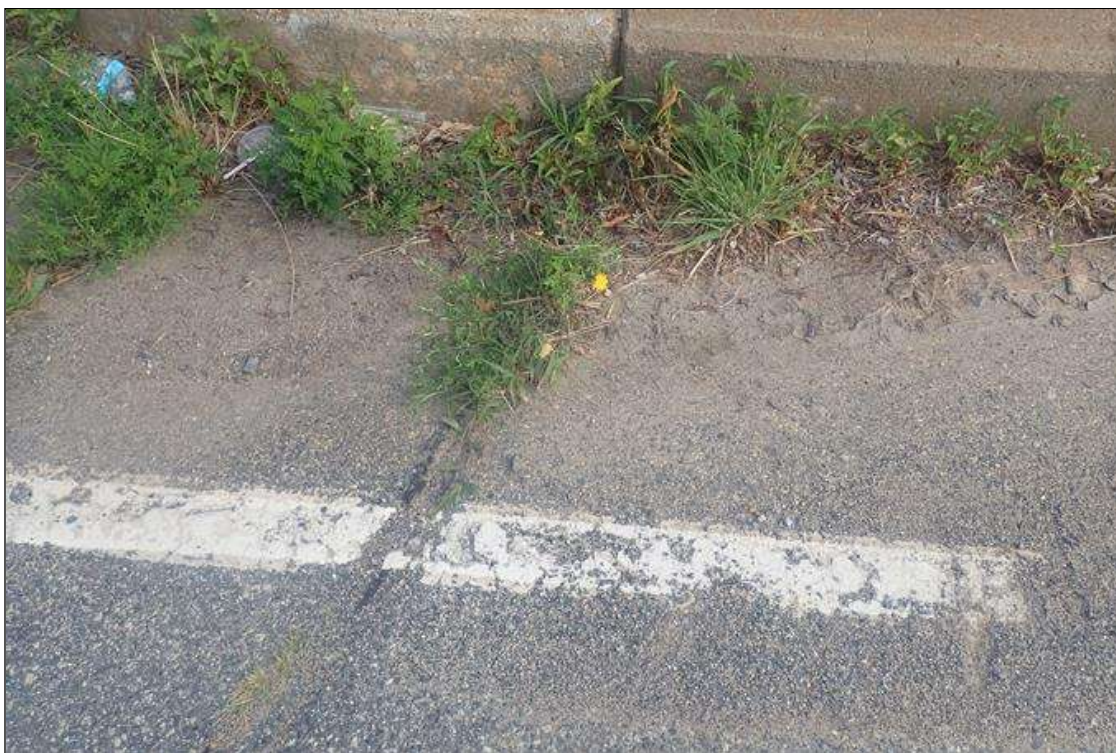
Span 4 Expansion Joint: DEBRIS IMPACTION AND VEGETATION GROWTH IN JOINT AT BOTH GUTTERLINES FOR FIRST 3 FEET
