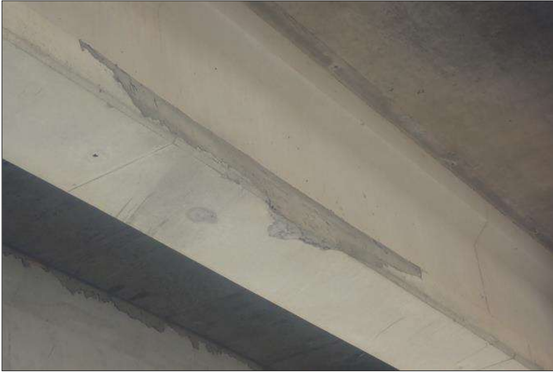
Span 3 Beam 3: PATCHED AREA THAT IS CRACKED ALONG BOTTOM FLANGE FROM IMPACT DAMAGE IN A 8 FEET LONG AREA OVER LEFT SOUTHBOUND LANE 02/16/2023 - IMPACT DAMAGE - OVERVIEW OF REPAIR AREA LOCATED OVER LEFT SOUTHBOUND LANE 25 FEET FROM BENT 3; DIMENSIONS ARE 8 FEET LONG ON NORTH SIDE OF BOTTOM FLANGE AND EXTEND APPROXIMATELY 10 INCHES UP 07/07/2023 no apparent change since supplemental inspection
