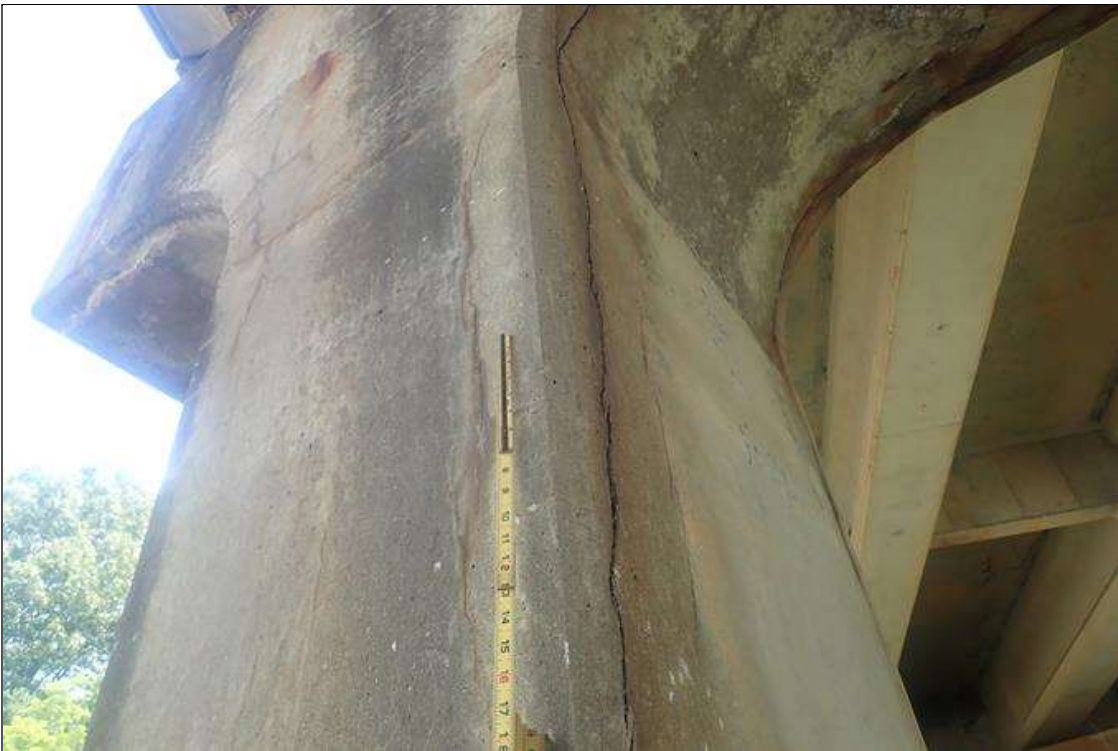
Bent 1 Pile 2: (PAR) VERTICAL CRACKS UP TO 1/8 INCH ALONG EDGES WITH DELAMINATIONS (UP TO 8 INCHES WIDE) FROM TOP DOWN 6 FEET WITH RUST STAINS ALL CORNERS.
