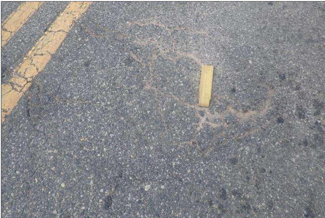
Span 1 Wearing Surface: SEVERAL AREAS TRANSVERSE AND MAP CRACKING / DETERIORATED ASPHALT WITH CRACKS UP TO 1/2 INCH, SOME AREAS SOUND DELAMINATED
