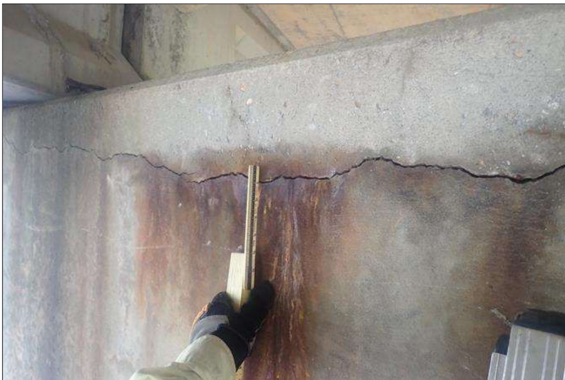
Bent 3 Cap 1: (PAR) 1/8 inch Horizontal crack on both faces of cap near top full length, with rust stains and some efflorescence buildup
