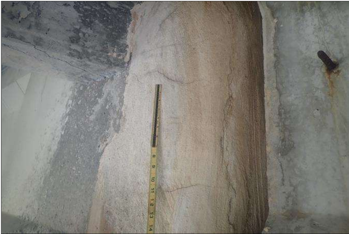
Span 2 Beam 2: Full height x 10 inch long patched area with cracks (up to 1/32 inch) in right side web at pier 2
