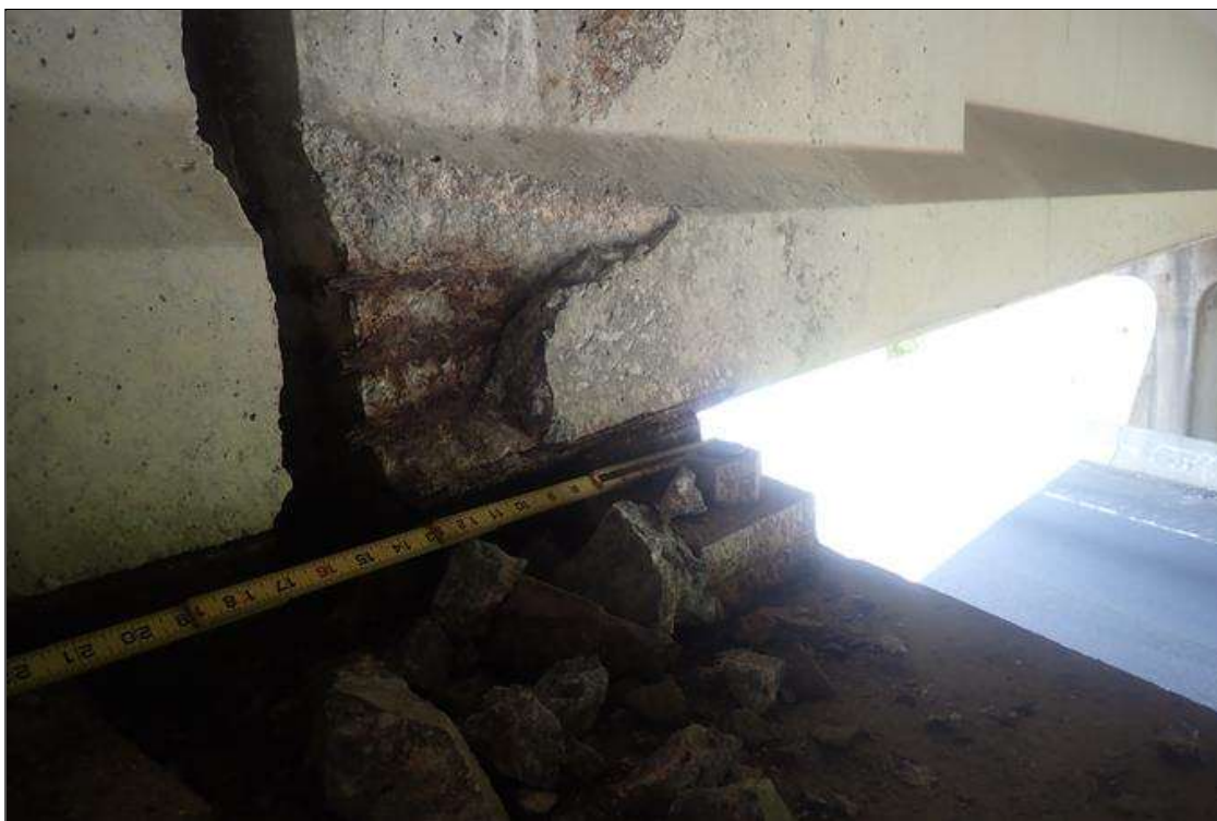
Span 2 Beam 3: (PAR) 16 inch x 9 inch x 2 inch deep spall with exposed rusted strands in left side bottom flange at pier 2
