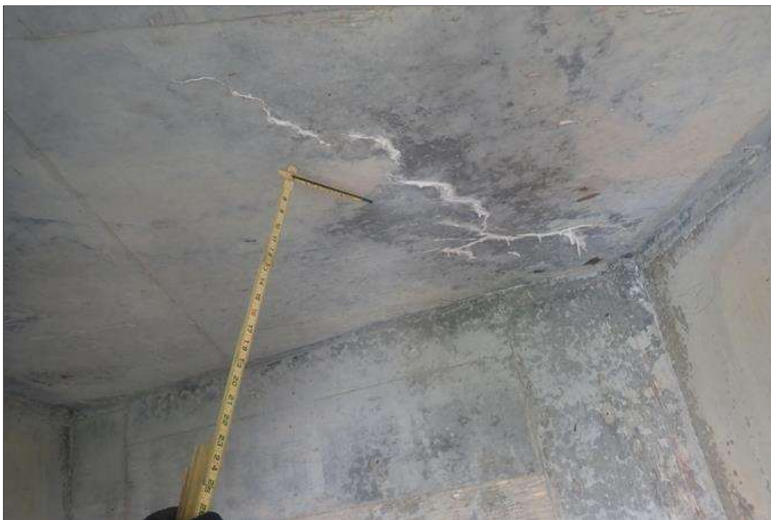
Span 1 Deck: (PAR) underside, bay 3, at end bent 1, diagonal crack (hairline x 5 feet) with efflorescence buildup
