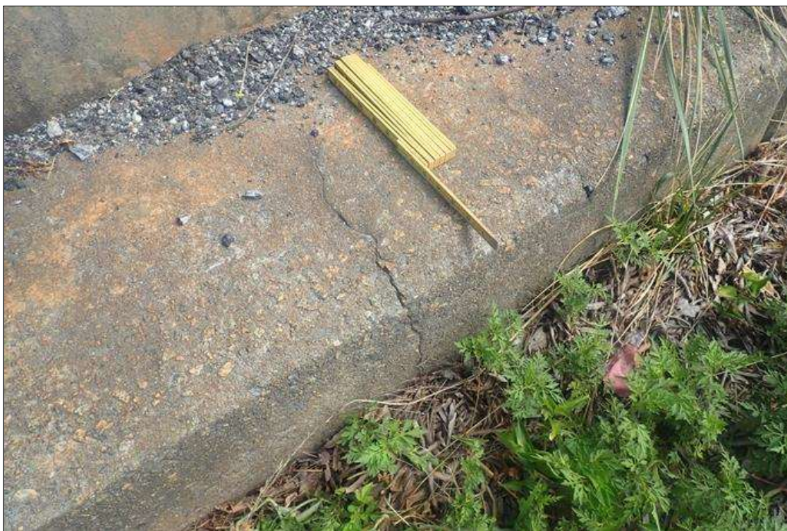
Span 1 Right Bridge Rail: curb, at end bent 1, transverse crack (1/16 inch x full width)
