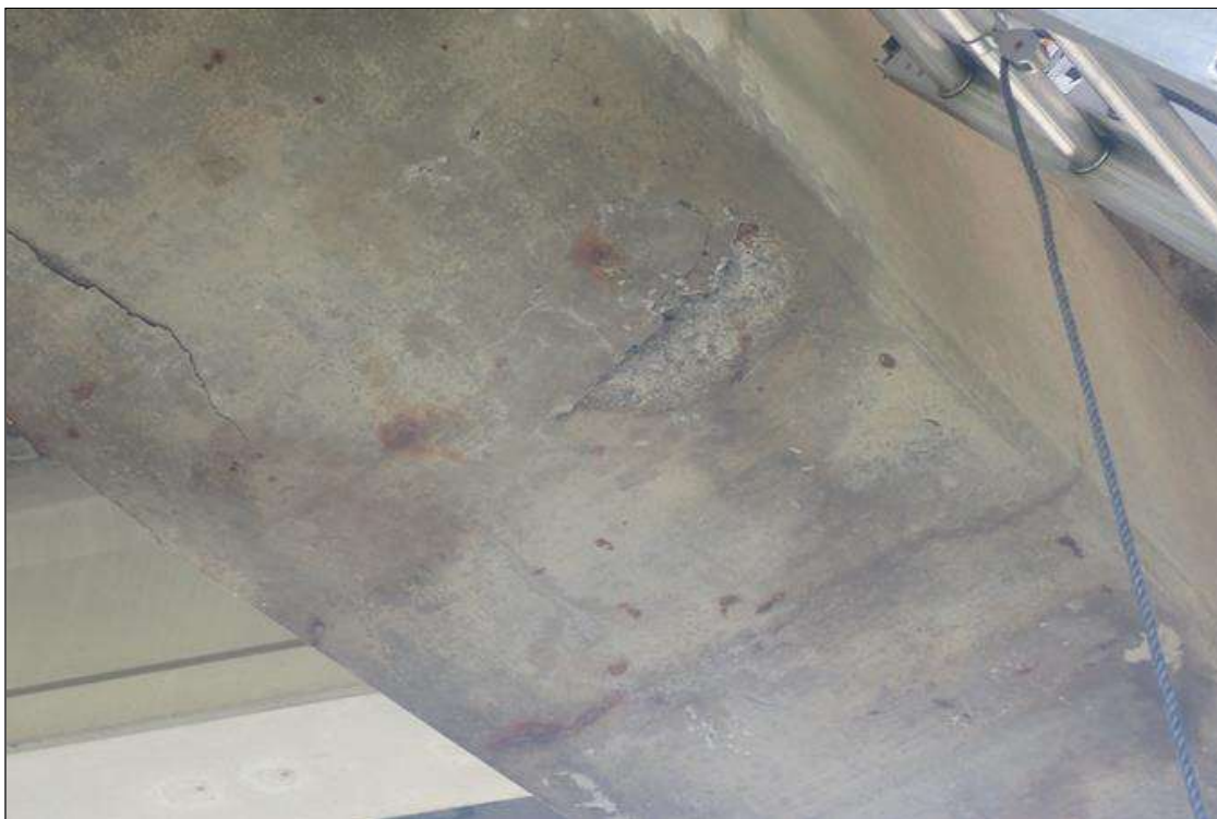
Bent 2 Cap 1: (PAR) underside of cap, longitudinal/transverse cracks (hairline up to 1/16 inch x full width x 12 feet) with rust stains and delamination/spall (up to full width x 1 inch deep)
