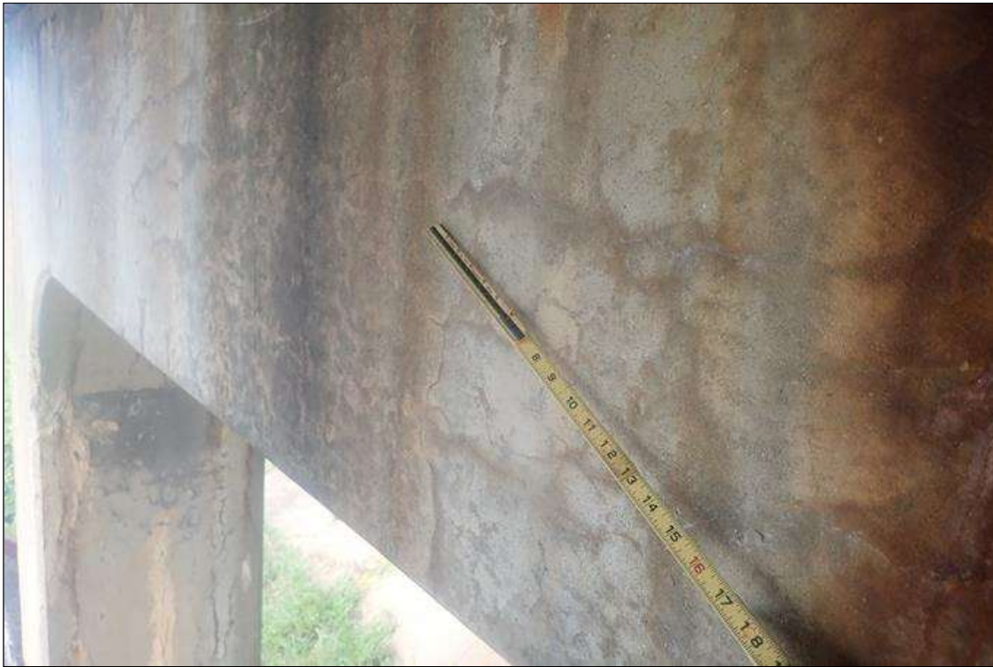
Bent 3 Cap 1: SCATTERED AREAS OF HAIRLINE MAP CRACKS WITH EFFLORESCENCE THROUGH OUT CAP
