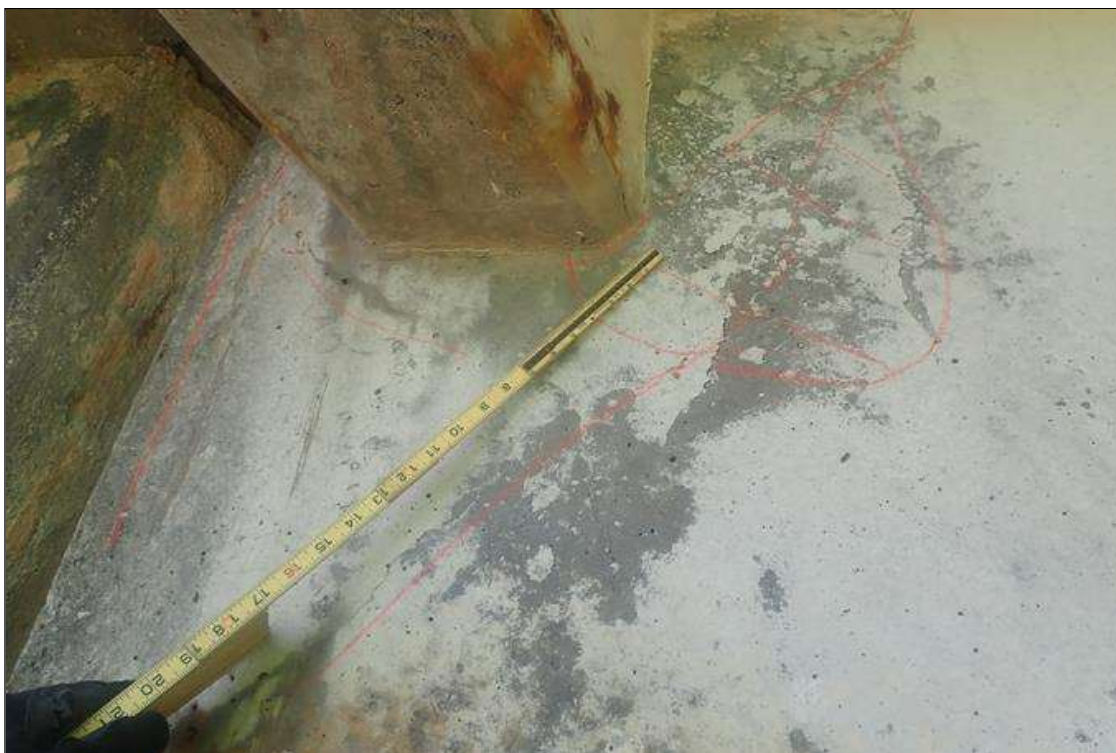
Span 4 Beam 4: (PAR) at bent 3, right face, web, vertical and diagonal crack (up to 0.01 inch x 4 feet) with delamination (12 inch x 16 inch)
