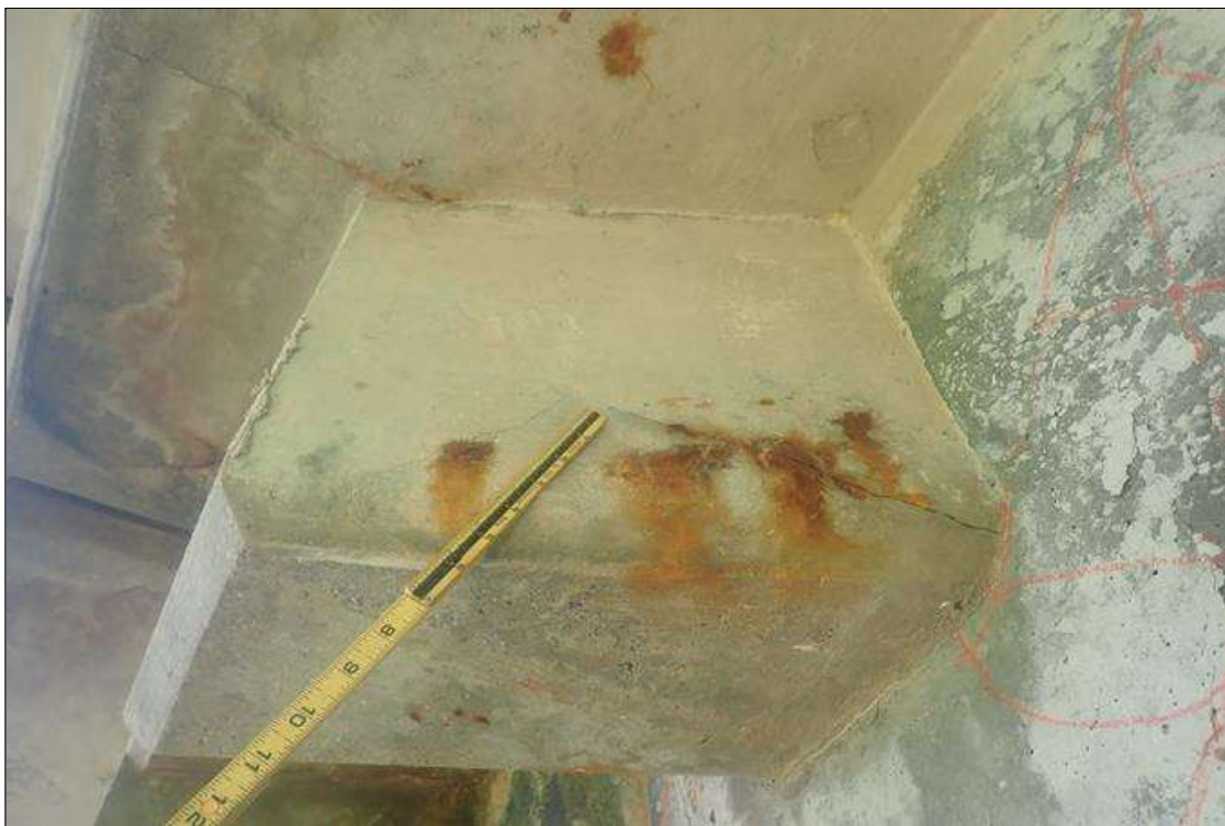
Span 4 Deck: (PAR) bent 3 end diaphragm, right overhang, longitudinal crack (1/32 inch x 12 inch) with rust stains
