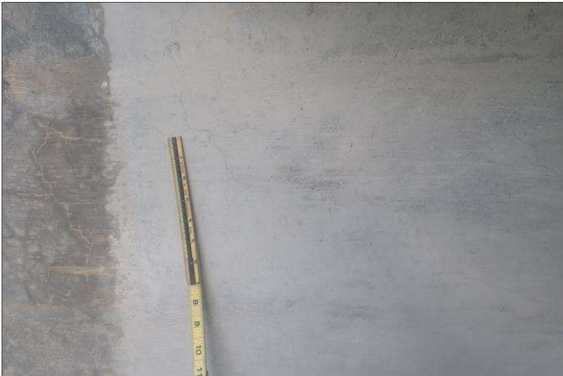
End Bent 1 Abutment: Area of hairline map cracks (4 feet x 2 feet) at east end of abutment
