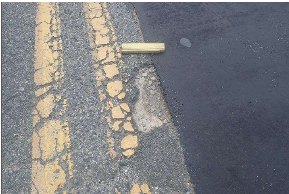
Span 2 Wearing Surface: multiple full depth potholes up to 15 inches wide x 8 inches long near centerline roadway and northbound lane
