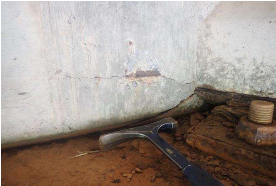
End Bent 1 Abutment: 4 inch long x 3 inch high x 1 inch deep spall with exposed rebar at right side of beam 2
