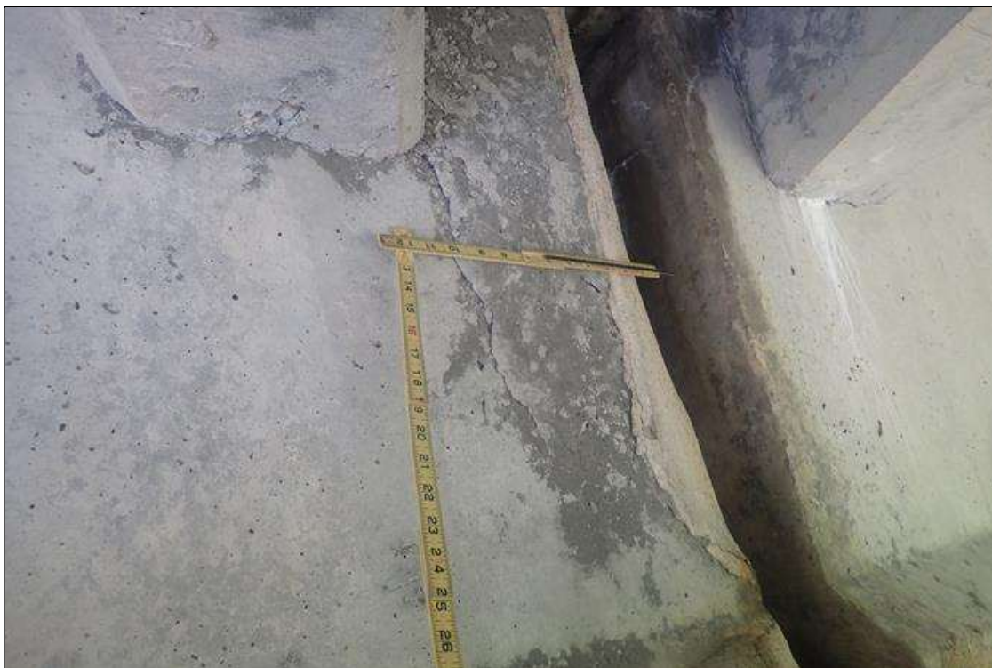
Span 2 Beam 2: at bent 1, web, left face, delamination (10 inch x full height)
