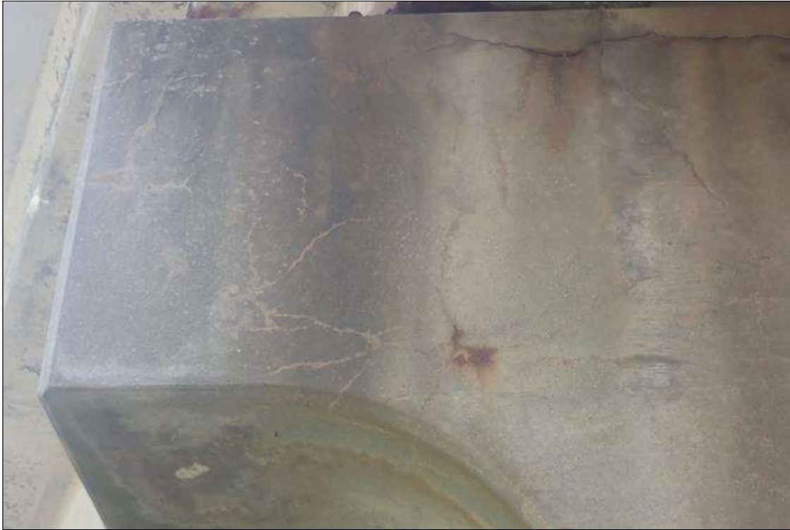
Bent 2 Cap 1: (PAR) north face, right end, map cracks (hairline x 3 feet x full height) with efflorescence and rust stains
