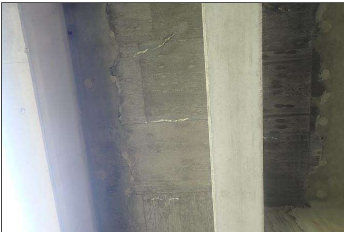
Span 3 Deck: underside, bays 1 and 2, transverse cracks (hairline x 6 feet) with efflorescence
