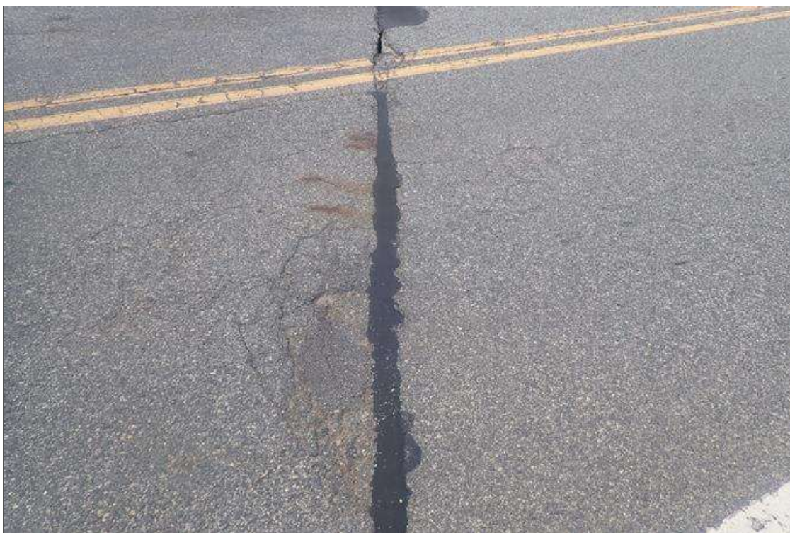
Span 3 Wearing Surface: northbound lane at bent 3 joint, sealed transverse crack (12 foot)
