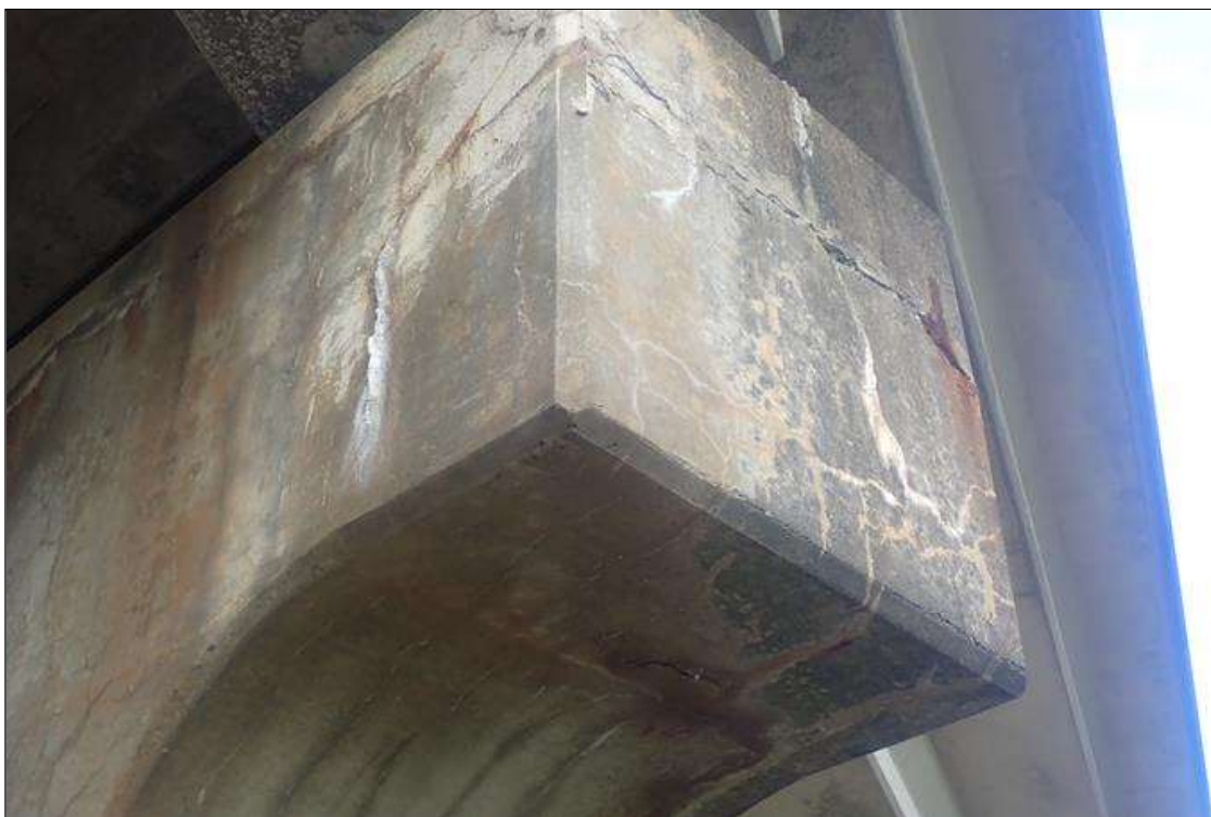
Bent 3 Cap 1: (PAR) both ends of cap, map cracks (hairline) with efflorescence buildup
