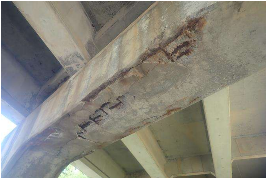
Bent 1 Cap 1: (PAR) SPALL AND DELAMINATION ALONG BOTTOM CAP BETWEEN COLUMNS 15 FEET LONG X FULL WIDTH X 3 INCHES DEEP WITH EXPOSED STEEL. EXPOSED STEEL HAS UP TO 1/8 INCH LOSS.
