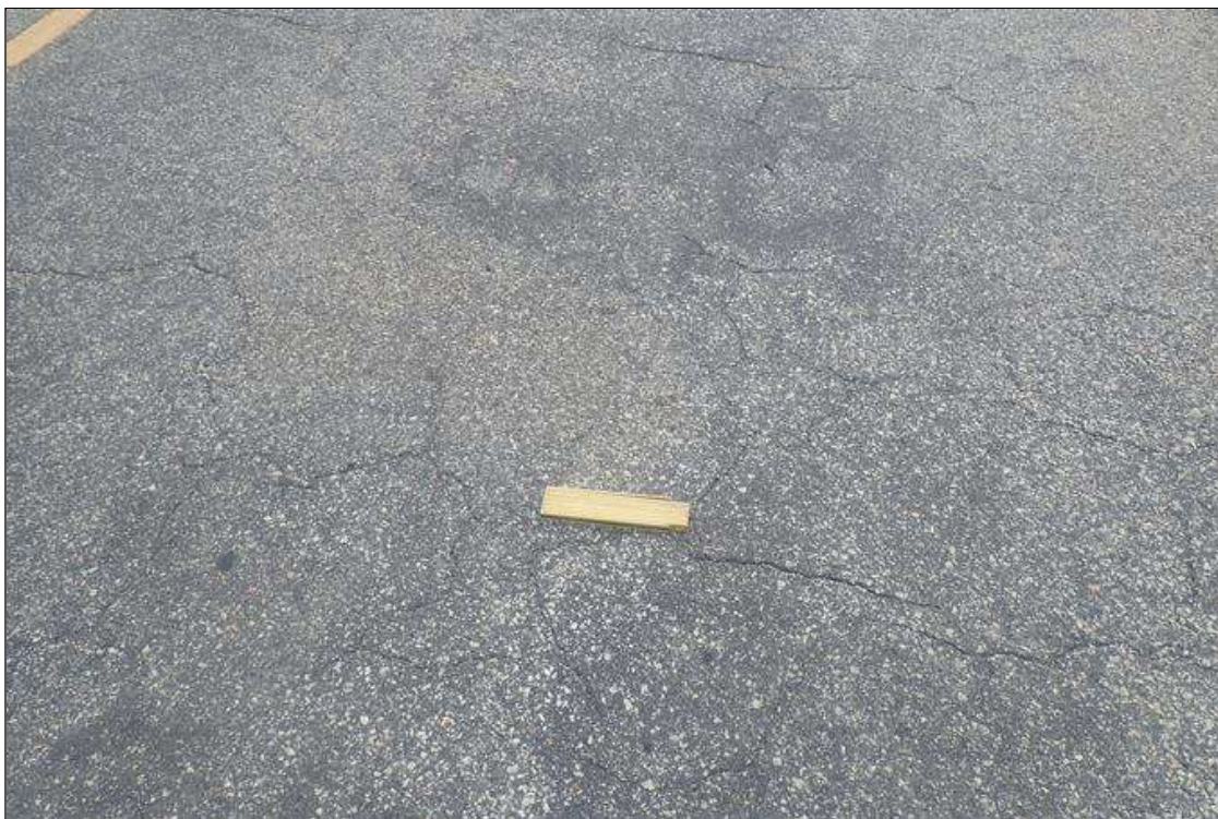
Span 3 Wearing Surface: throughout southbound lane, and at random in northbound lane, longitudinal/map cracks (up to 1/2 inch), some with rust stains, some areas sound delaminated
