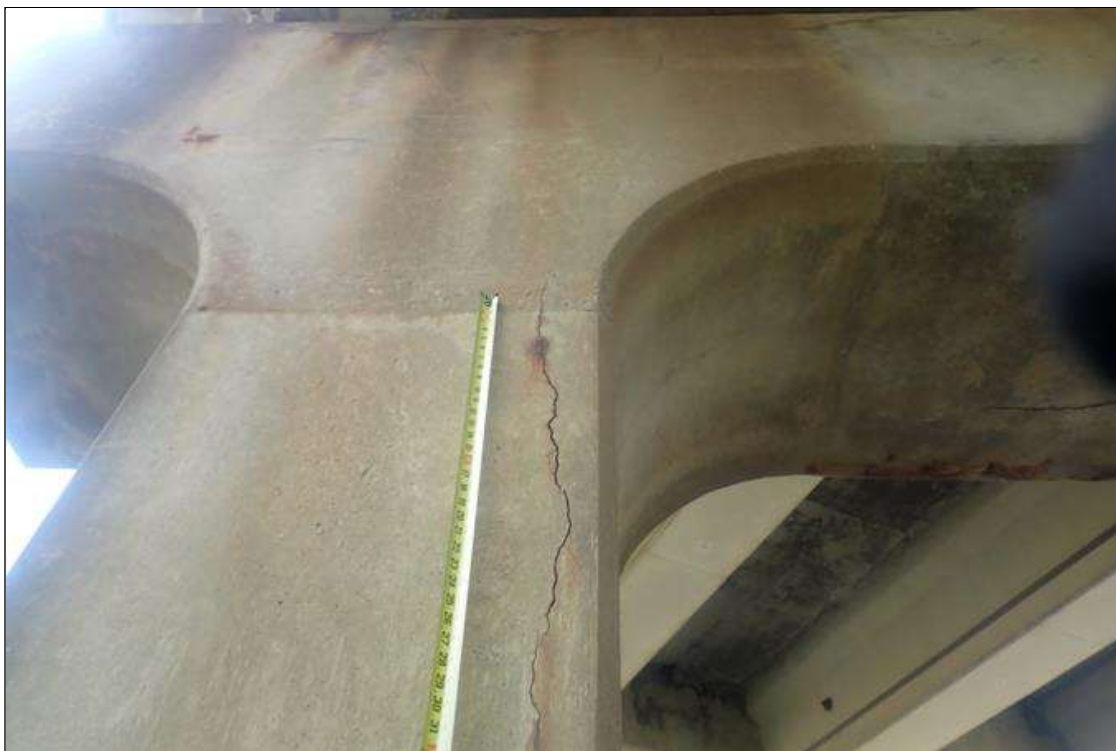
Bent 2 Pile 2: (PAR) 1/8 inch vertical crack 4 feet long with rust stains on northwest corner near top
