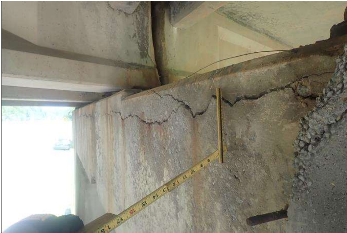
Bent 1 Cap 1: (PAR) HORIZONTAL CRACKING UP TO 1/4 INCH WITH SEVERAL AREAS OF DELAMINATIONS AND RUST STAINS WHICH EXTENDS 6 INCHES ON TOP OF CAP ALONG LENGTH OF BOTH FACES.
