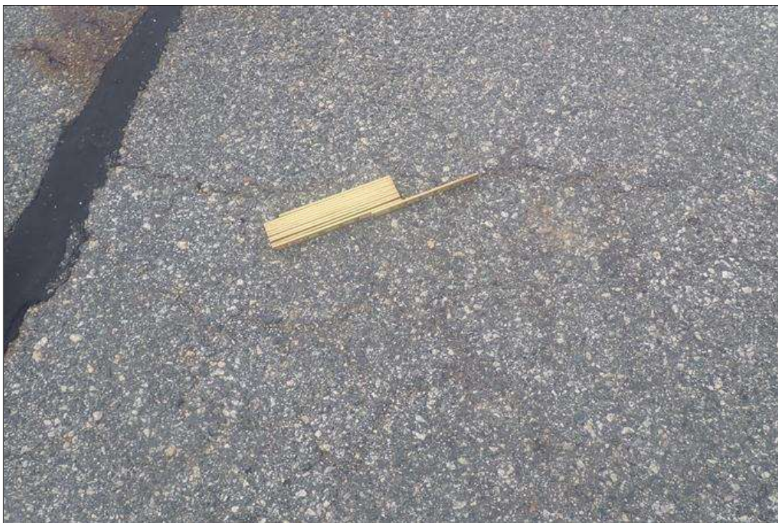
Span 4 Wearing Surface: northbound lane, at random, areas of map cracks (up to 1/8 inch x 2 feet x 3 feet), some areas sound delaminated
