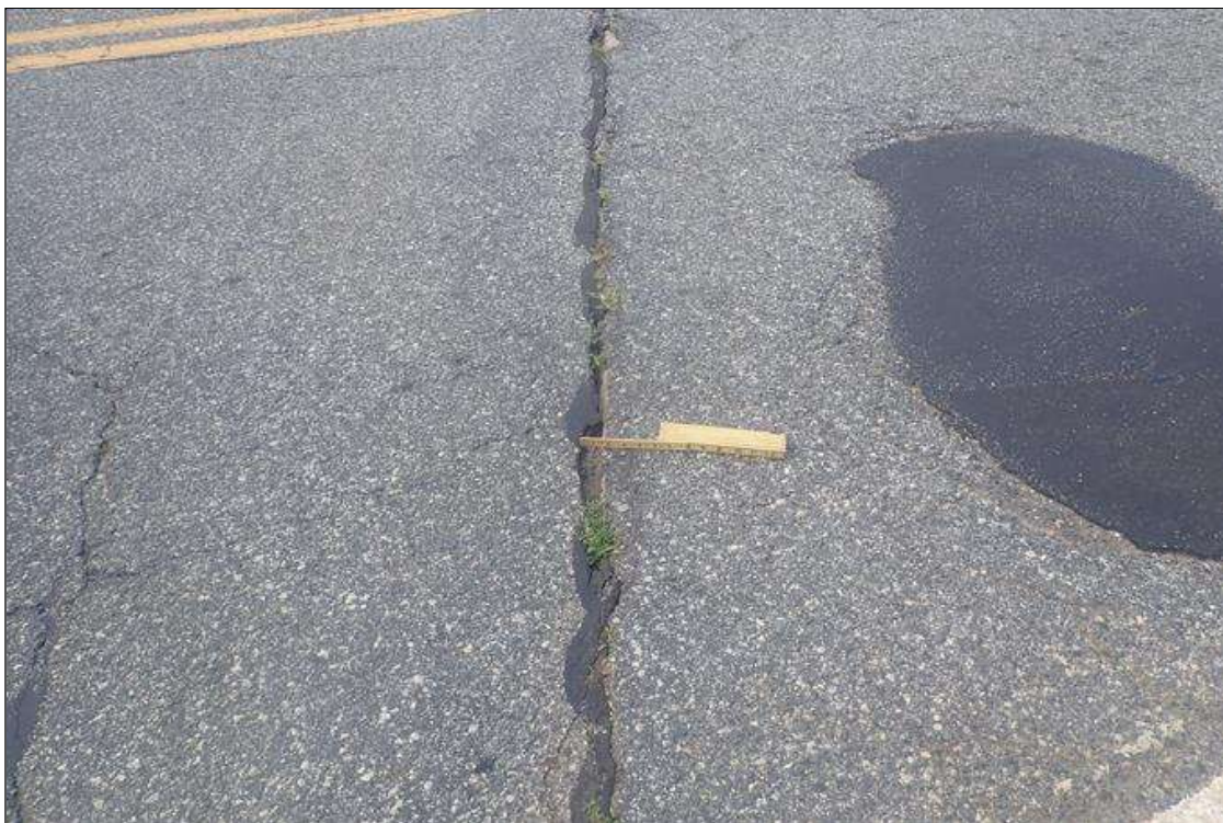
Span 1 Wearing Surface: Full width transverse cracks up to 1.5 inch at abutment 1 with failed sealant
