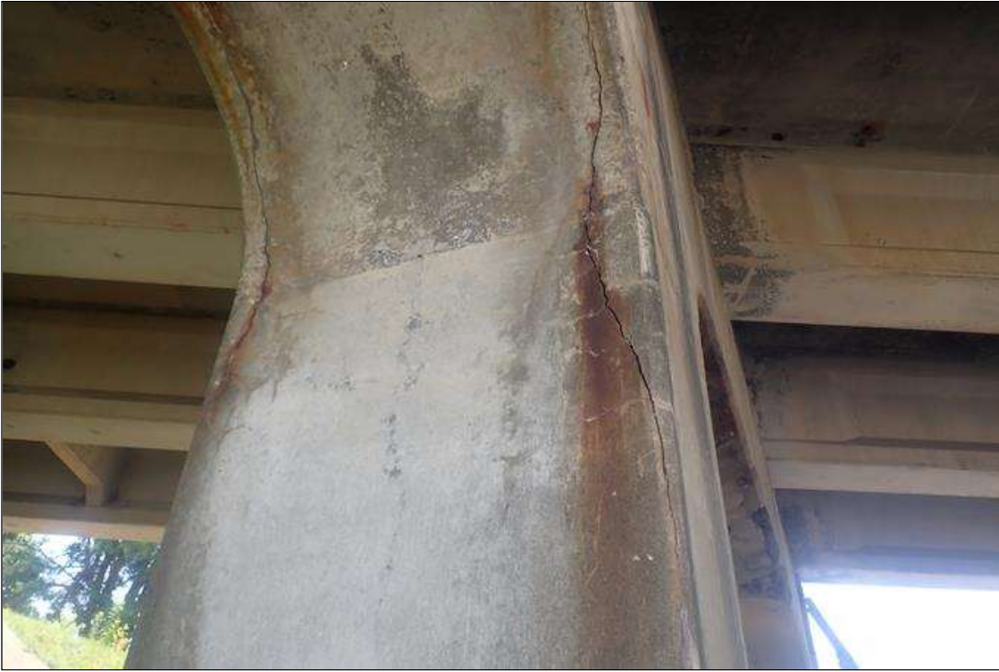
Bent 1 Pile 2: (PAR) VERTICAL CRACKS UP TO 1/8 INCH ALONG EDGES WITH DELAMINATIONS (UP TO 8 INCHES WIDE) FROM TOP DOWN 6 FEET WITH RUST STAINS ALL CORNERS.
