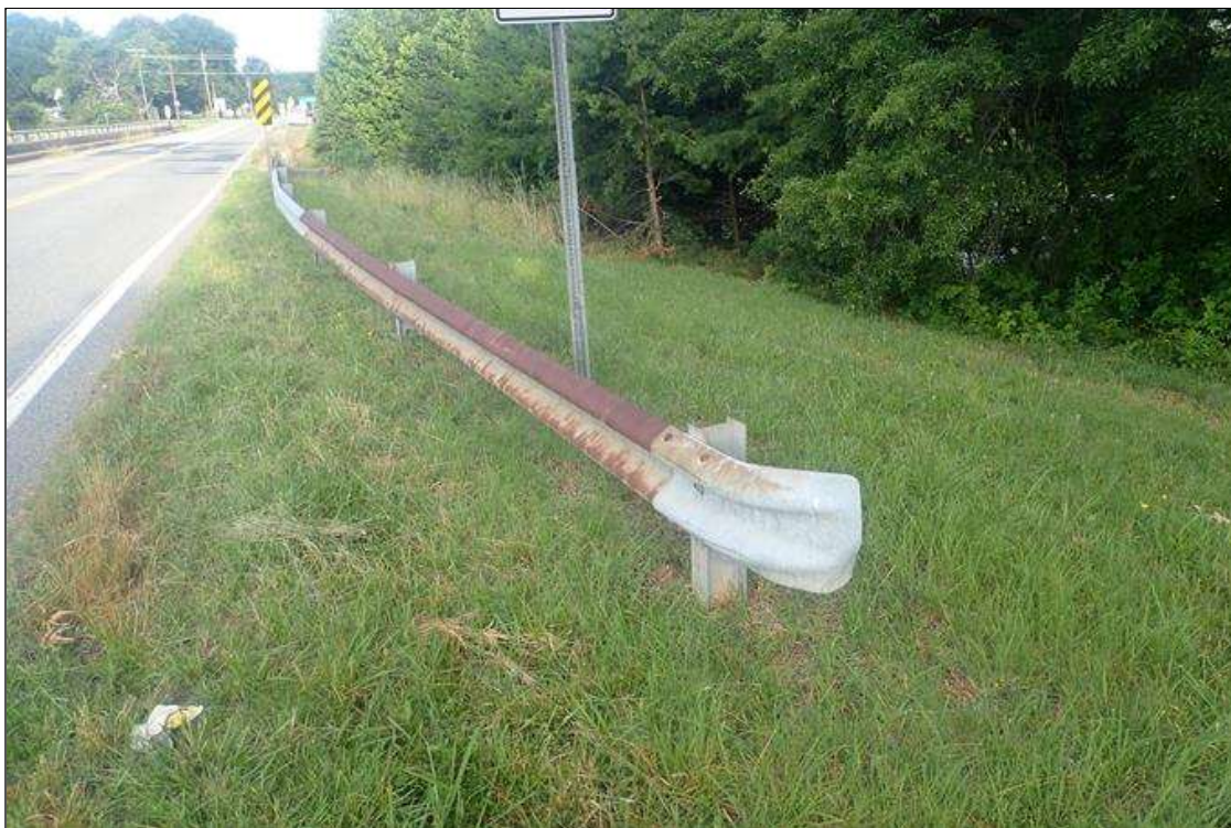
southeast guardrail and termination
