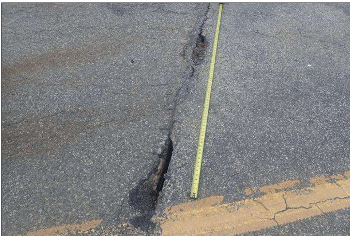
Span 3 Expansion Joint: southbound lane, joint material missing (7 feet)
