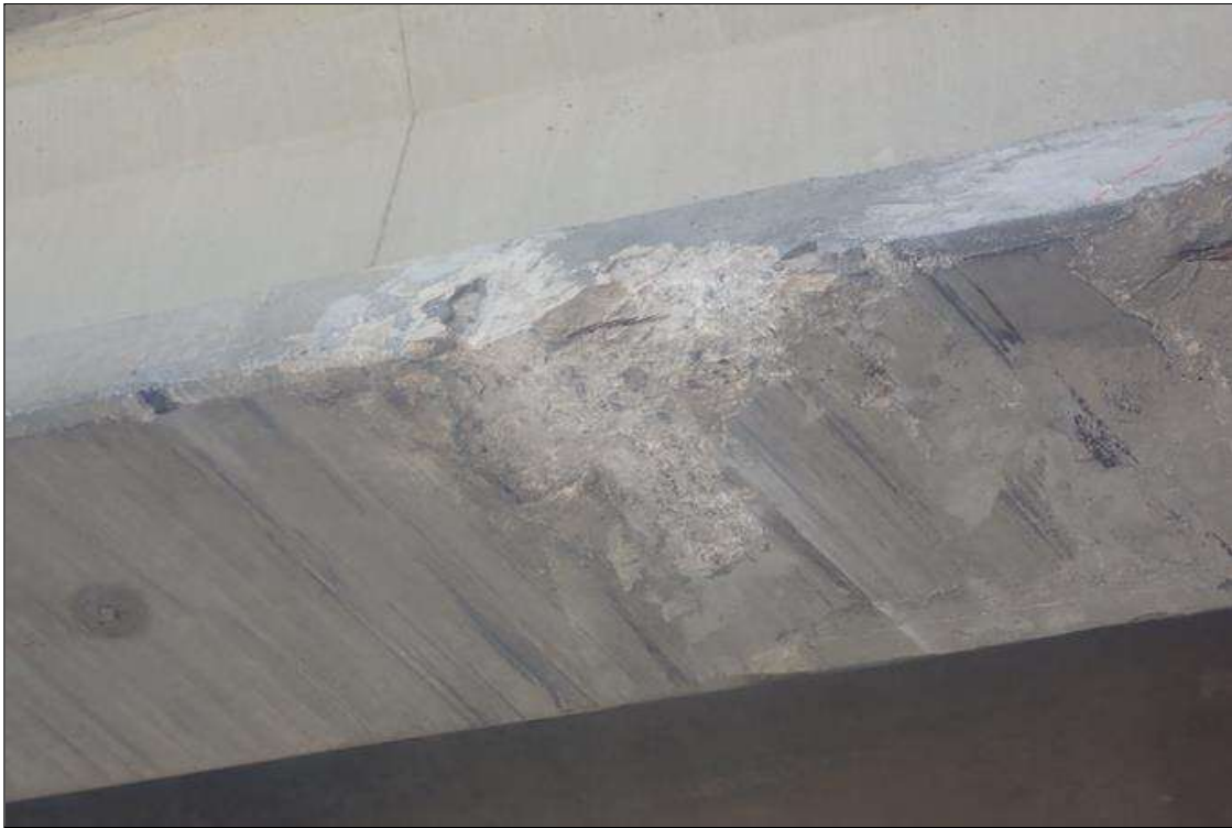
Span 3 Beam 4: (PAR) IMPACT DAMAGE - LOCATED 20 FEET FROM BENT 3; DIMENSIONS ARE 1.333 FEET LONG X 22 INCHES WIDE X 4 INCHES DEEP WITH EXPOSED RUSTED STRAND, ON NORTH EDGE OF BOTTOM FLANGE AND CONTINUING ACROSS FULL WIDTH OF BOTTOM FLANGE.
