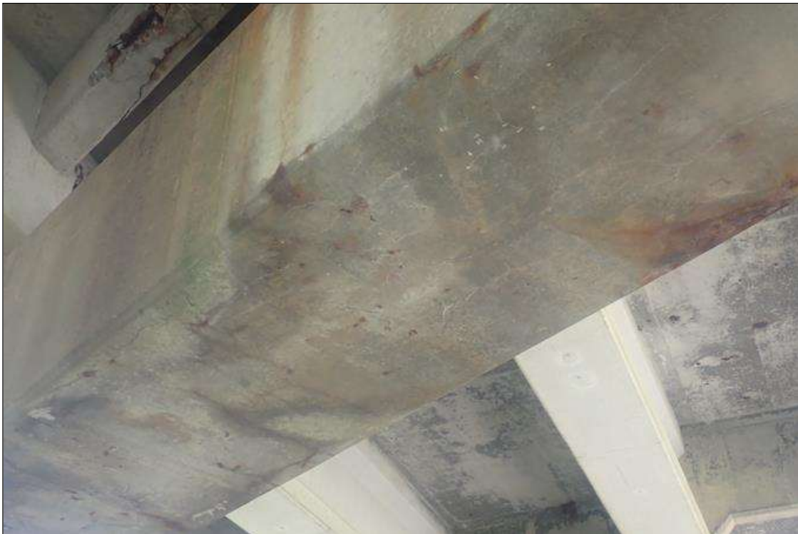
Bent 2 Cap 1: (PAR) underside of cap, longitudinal/transverse cracks (hairline up to 1/16 inch x full width x 12 feet) with rust stains and delamination/spall (up to full width x 1 inch deep)
