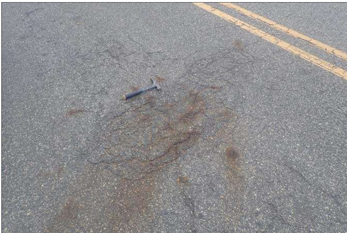
Span 4 Wearing Surface: northbound lane, 10 feet from end bent 2, map cracks (up to 1/2 inch x 7 feet x 4 feet) with rust stains, area sounds delaminated
