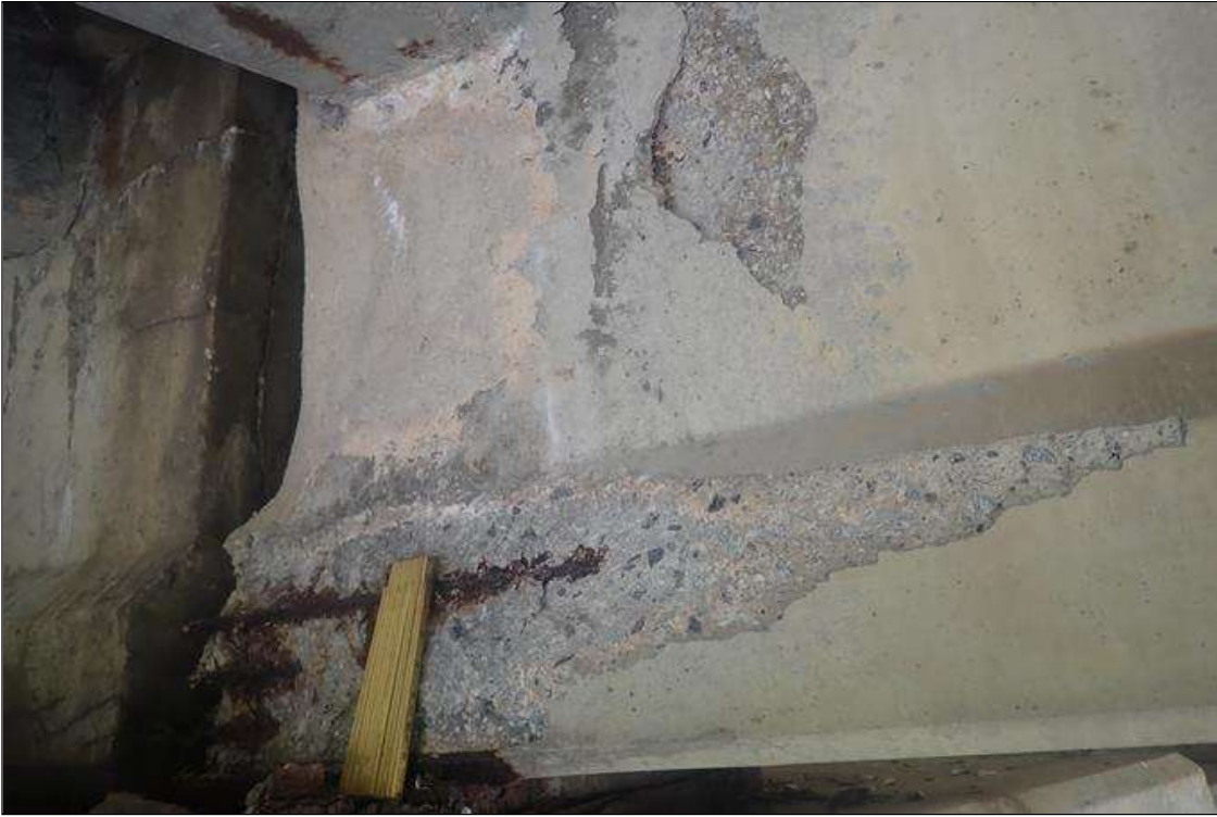
Span 2 Beam 2: (PAR) at bent 1, right face, spall/delamination (3 feet x full height) with exposed rusted strands and rebar, with partial patch in web
