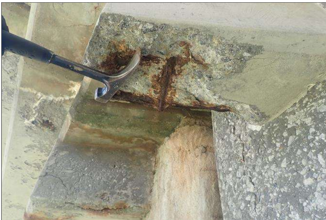
Span 3 Deck: bent 2 end diaphragm, right overhang, spall (12 inch x 8 inch x 2 inch deep)
