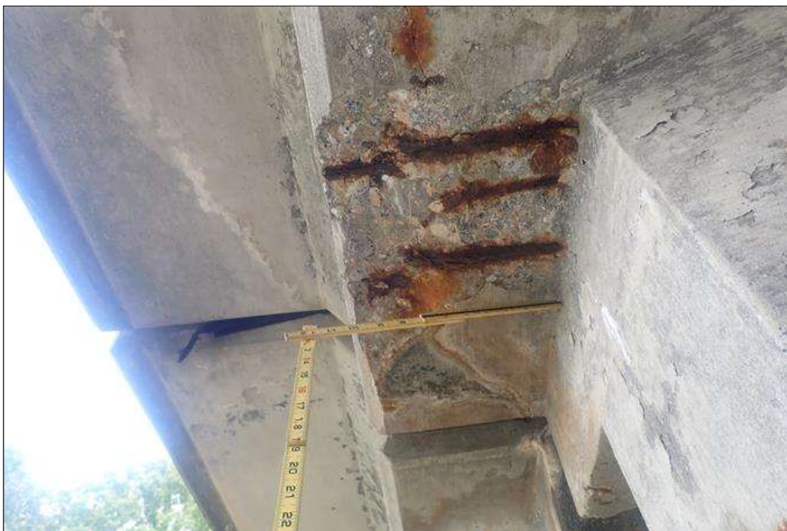
Span 2 Deck: (PAR) right overhang, at bent 1, spall (10 inch x 12 inch x 1.5 inch deep) with exposed rusted rebar
