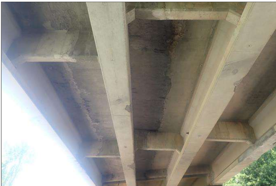
Span 3 Deck: FULL LENGTH SOUND PATCHED AREAS 4 FEET WIDE UNDERSIDE OF DECK BAYS 1 AND 2 ADJACENT TO BEAM 2.
