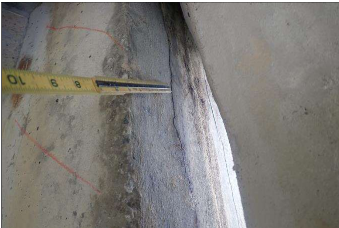
Span 1 Beam 1: (PAR) at bent 1, web, right face, delamination (12 inch x full height) with rust stains; end face, (2) vertical cracks (0.06 inch x full height)
