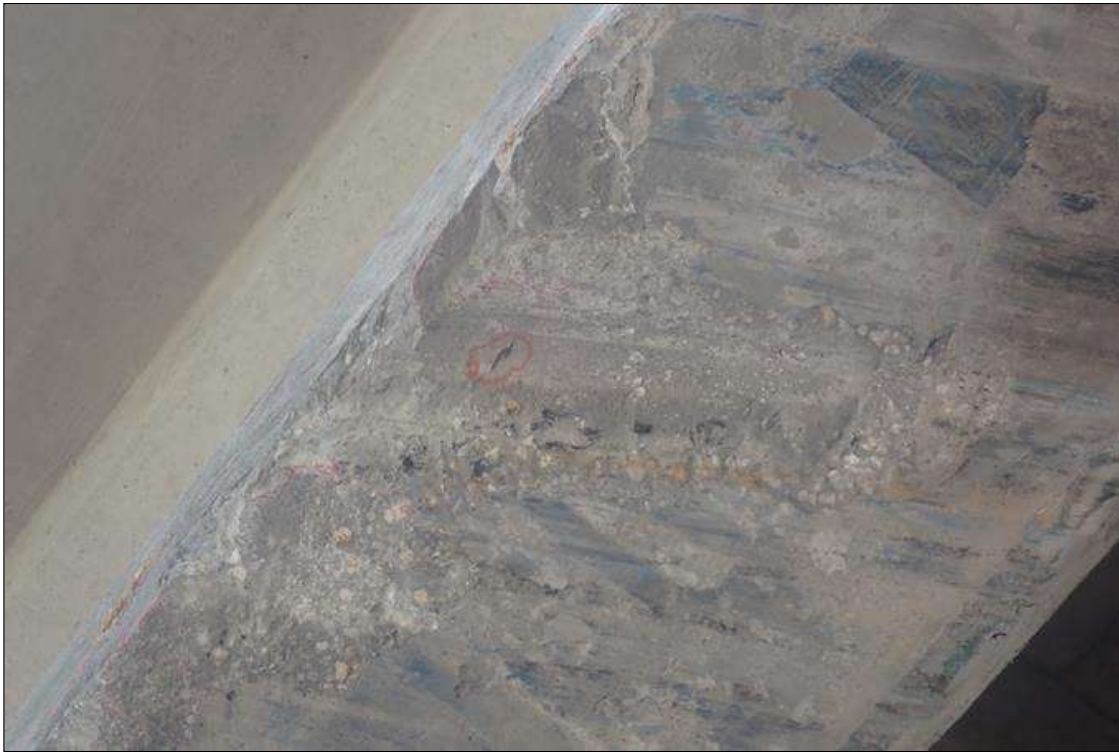
Span 3 Beam 4: (PAR) 8 INCHES X 8 INCHES X 1 INCH DEEP SPALL DUE TO IMPACT ON EAST SIDE OF BOTTOM FLANGE OVER left southbound TRAVEL LANE ADJACENT TO SOUND PATCH - 02/16/2023 - IMPACT DAMAGE - LOCATED 14 FEET 8 INCHES FROM BENT 3 OVER LEFT TRAVEL LANE - DIMENSIONS ARE 1-1/2 FEET X 8 INCHES HIGH X 1-1/2 INCHES DEEP WITH ONE (1) STRAND OF EXPOSED REBAR SHOWING ON BOTTOM OF GIRDER - 07/07/2023 defect is over right southbound lane; no apparent change from supplemental inspection
