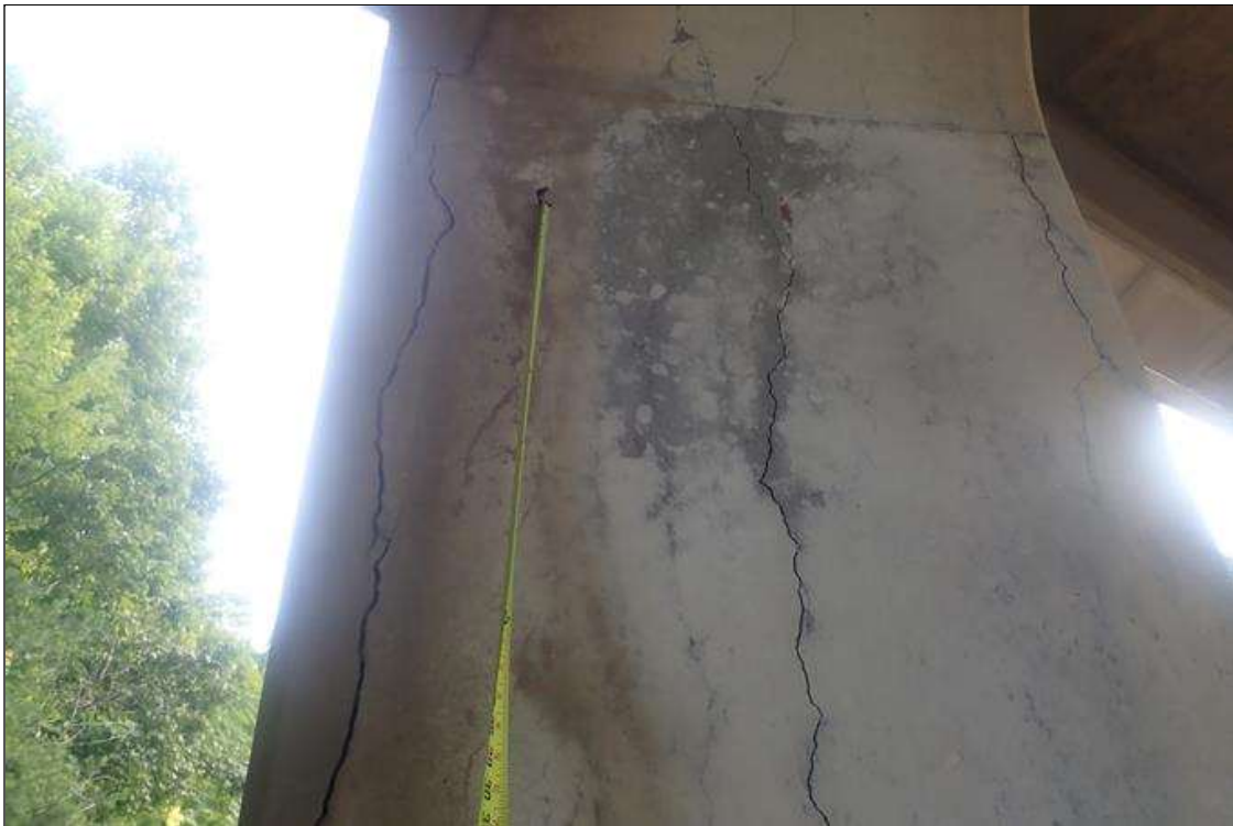
Bent 3 Pile 2: (PAR) VERTICAL CRACKING UP TO 3/16 INCH AND DELAMINATION UP TO 6 INCH WIDE ON ALL 4 SIDES WITH SOME OF CRACKS SEALED OVER BUT STILL CRACKED THROUGH TOP TO BOTTOM WITH RUST STAINS.
