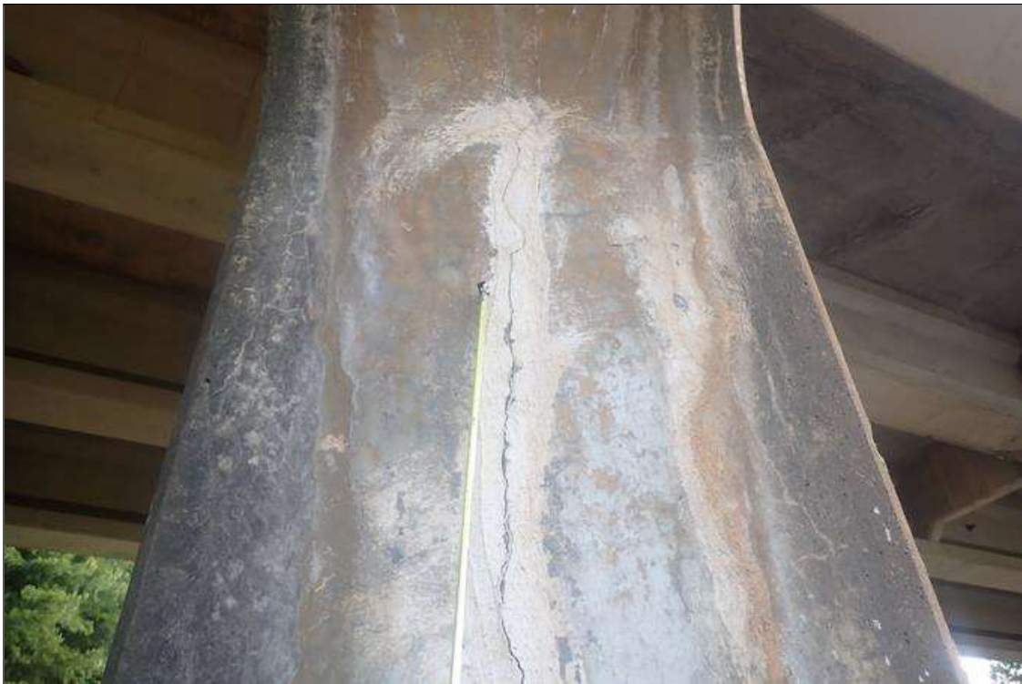
Bent 3 Pile 1: (PAR) VERTICAL CRACKING UP TO 1/8 INCH AND DELAMINATION UP TO 6 INCH WIDE ON ALL 4 SIDES WITH SOME OF CRACKS SEALED OVER BUT STILL CRACKED THROUGH TOP TO BOTTOM WITH RUST STAINS.
