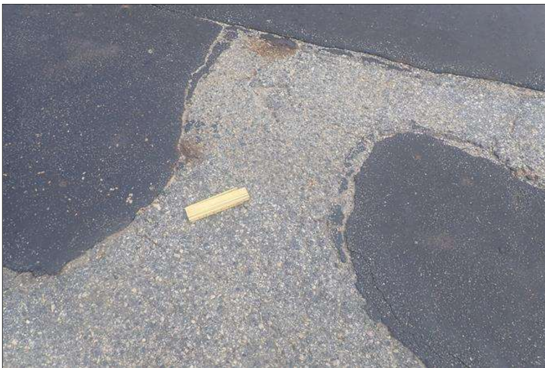
Span 2 Wearing Surface: SEVERAL AREAS TRANSVERSE AND MAP CRACKING / DETERIORATED ASPHALT WITH CRACKS UP TO 1/2 INCH, SOME WITH RUST STAINS, SOME AREAS DELAMINATED
