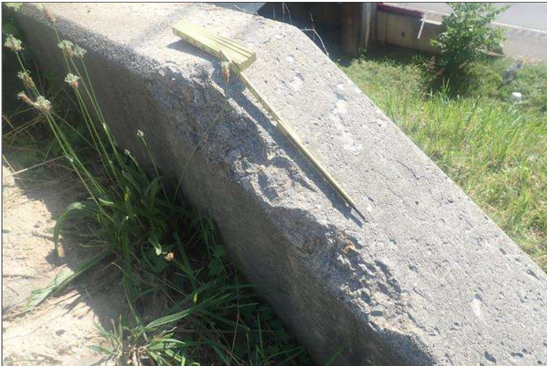
northwest wingwall, top corner, spall (2 foot x 3 inch x 1.5 inch deep)
