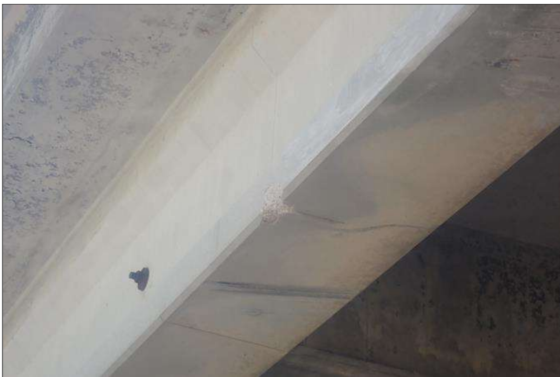
Span 2 Beam 4: 2 CHIPPED AREAS ALONG BOTTOM EDGES OF FLANGE UP TO 6 INCH X 6 INCH X 3/4 INCH DEEP FROM IMPACT DAMAGE AT MIDSPAN.
