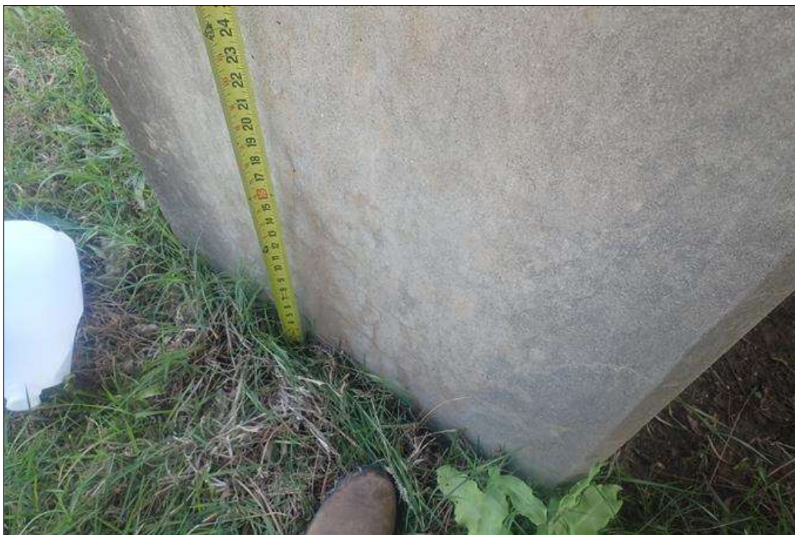
Bent 2 Pile 1: at ground, all faces, map cracks (hairline x 2 feet high)
