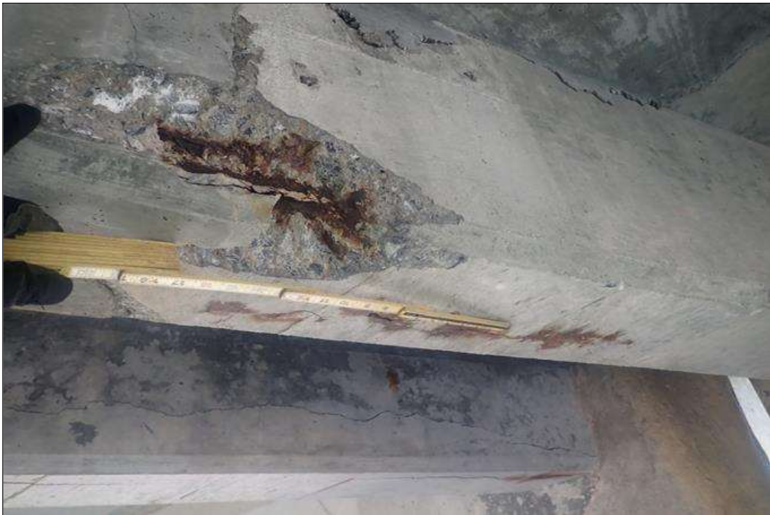
Span 3 Deck: (PAR) bent 2 end diaphragm, bay 1, longitudinal crack (1/16 inch x 3 feet) with rust stains and spall (16 inch x 6 inch x 2 inch deep) with exposed rusted rebar
