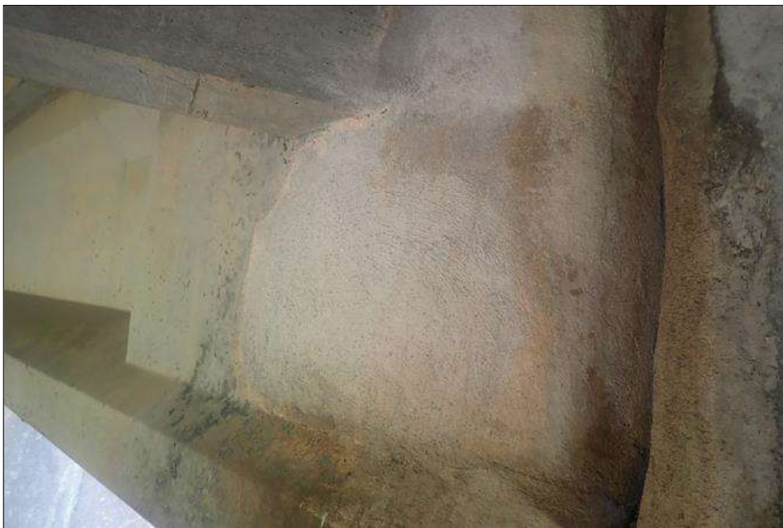
Span 4 Beam 4: FULL HEIGHT X 3 FOOT LONG PATCHED AREA THAT IS SOUND ON LEFT SIDE OF WEB OVER PIER 3.
