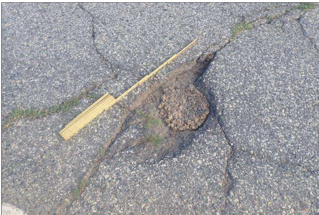
north approach asphalt, at bridge, transverse/map cracks (up to 1/2 inch); southbound lane, pothole (2 feet x 1 foot x 2 inch deep)
