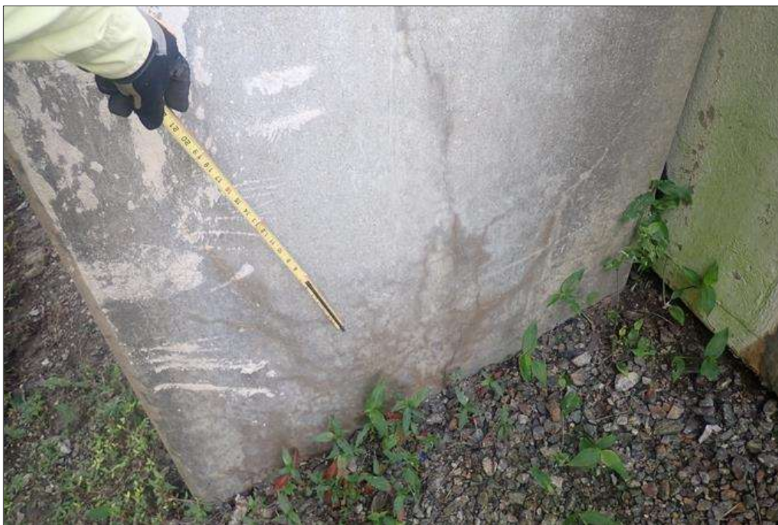
Bent 1 Pile 2: at ground, east and west faces, map cracks (hairline x 2 feet x 3 feet)
