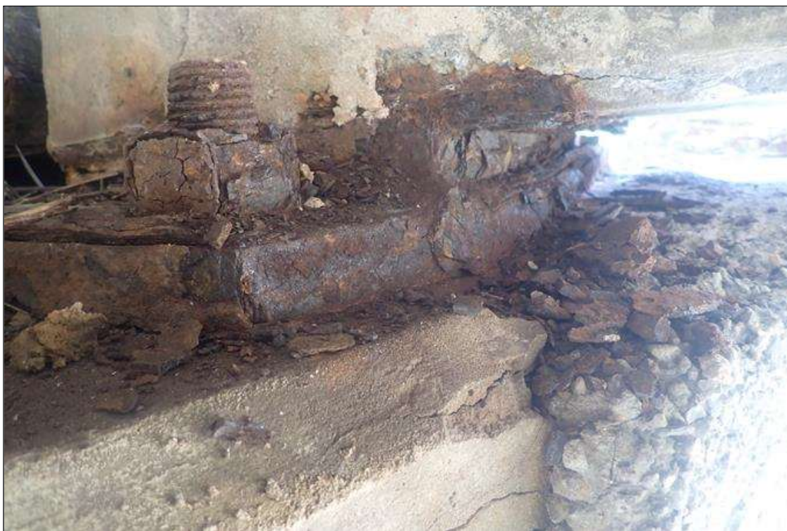
Span 2 Beam 1 - Near Bearing 1: rust scale/pack rust
