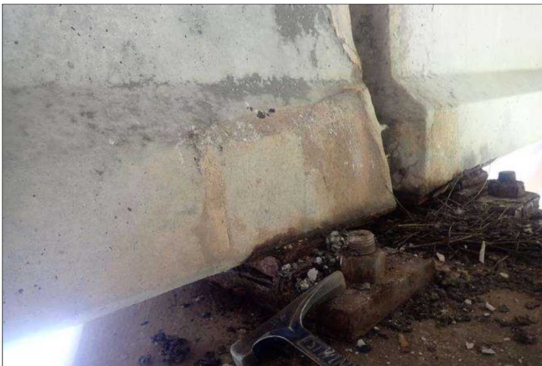
Span 2 Beam 2: FULL HEIGHT X 1.5 FOOT LONG PATCHED AREA ON BOTH SIDES OF BOTTOM FLANGE AND WEB OVER PIER 1.
