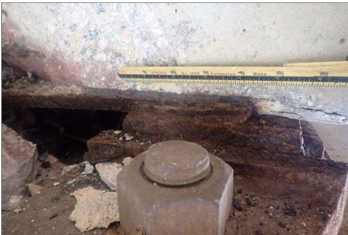
Span 3 Beam 3 - Far Bearing 3: beam installed with 4 inches of sole plate on bearing plate; no signs of distress
