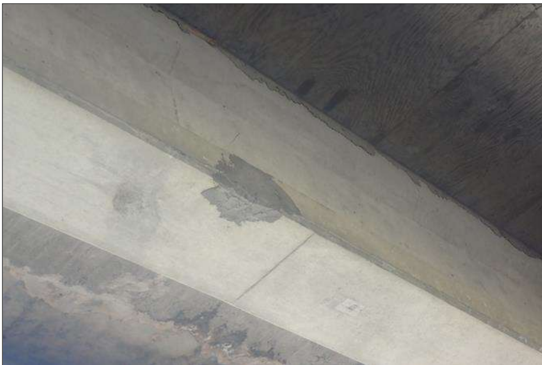
Span 3 Beam 2: (PAR) PATCHED AREA - LOCATED 25 FEET FROM BENT 3; 1 FOOT LONG X 8 INCHES HIGH, WITH MAP CRACKS UP TO APPROXIMATELY 1/32 INCH, POTENTIALLY DELAMINATED, OVER LEFT HAND SOUTHBOUND LANE
