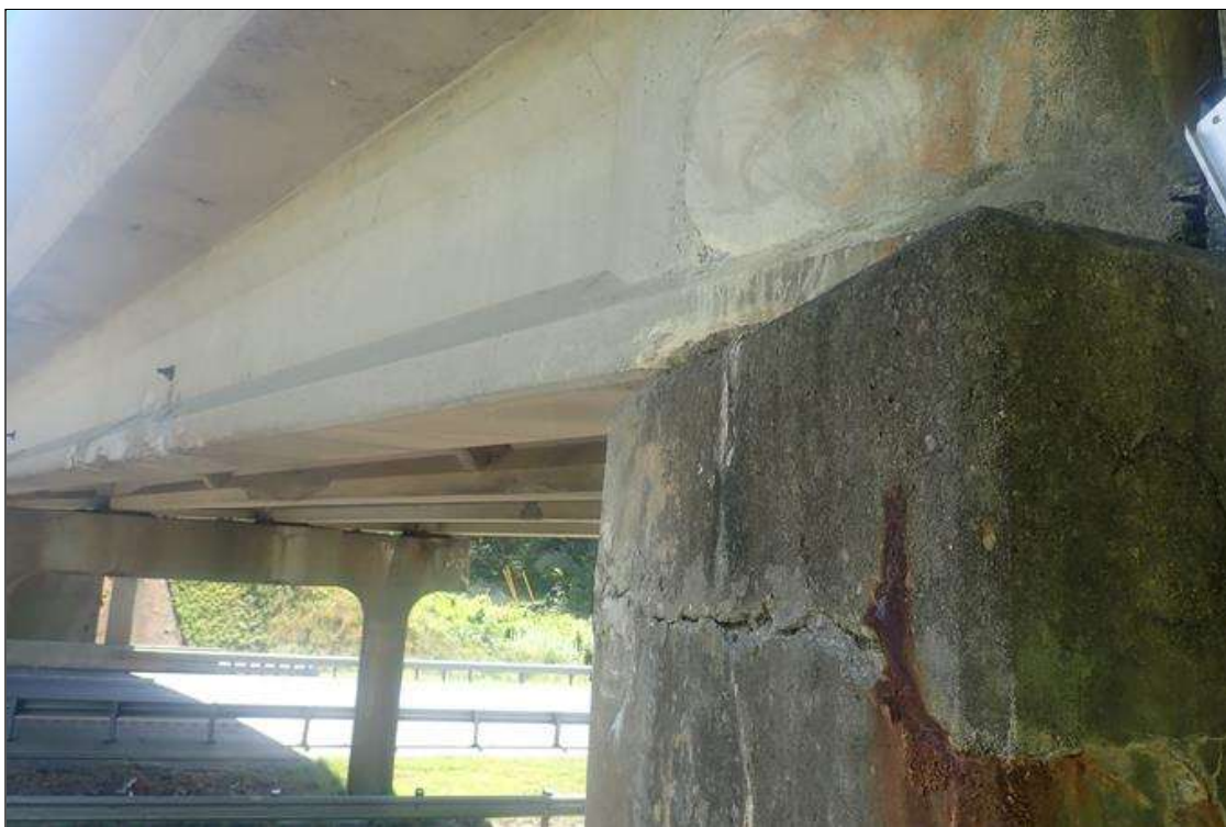
Bent 3 Cap 1: NORTH FACE OF CAP AT TOP, FULL WIDTH X 1.5 FOOT HIGH PATCHED AREA THAT HAS 2.5 INCHES OF EXPOSED REBAR
