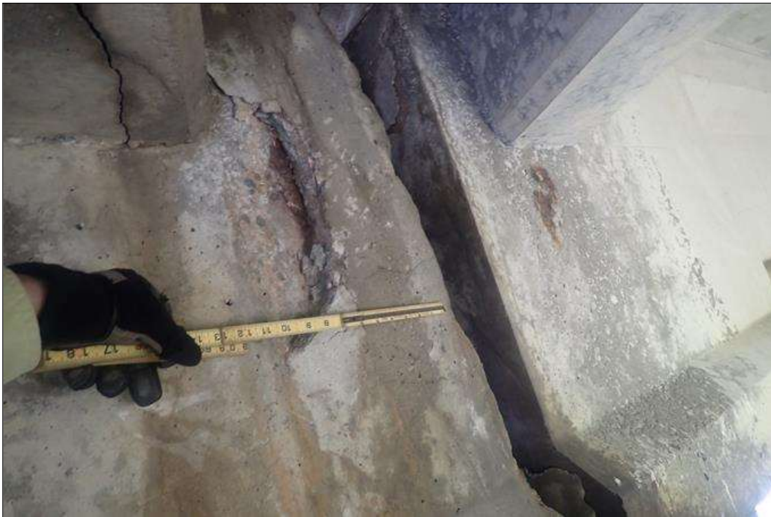
Span 2 Beam 4: (PAR) at bent 1, end of web, spall/delamination (30 inch high x full width x 2 inch deep) with exposed rusted rebar (up to 1/8 inch loss), extends along face of web (up to 10 inch)
