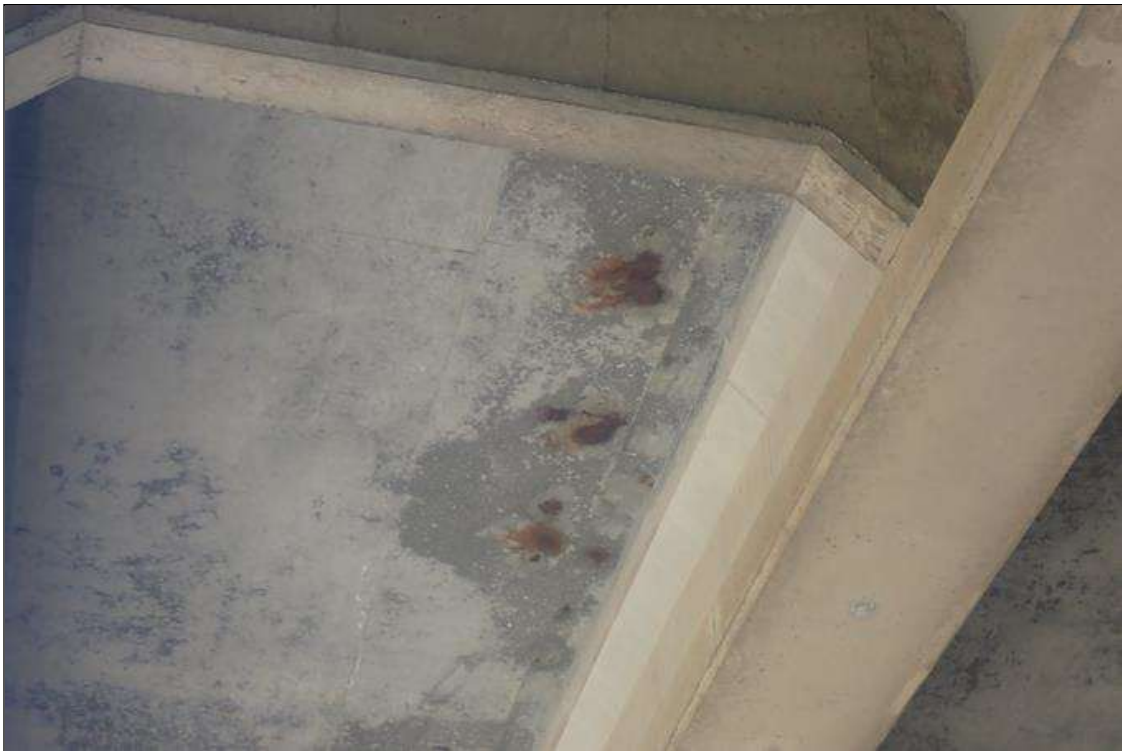
Span 2 Deck: (PAR) underside, at random, areas of transverse/map cracks (hairline) with rust stains
