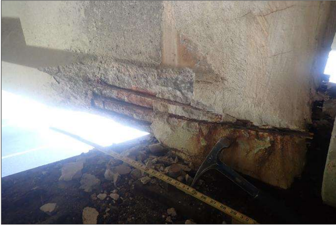
Span 2 Beam 2: (PAR) at bent 2, right face, bottom flange, spall (3.5 feet x 11 inch x 2 inch deep) with (2) broken strands and (1) rusted strand; similar left face
