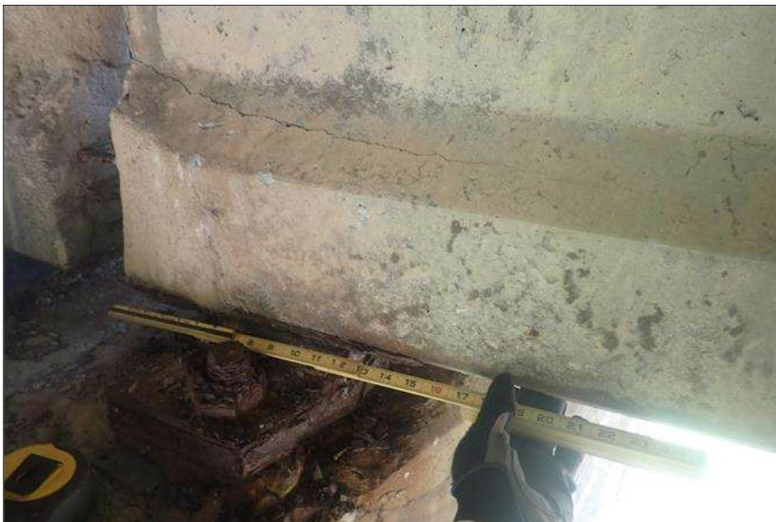
Span 3 Beam 1: at bent 2, right side, bottom flange, previous patch (6 inch x 6 inch) with delamination (2 feet x 8 inch)
