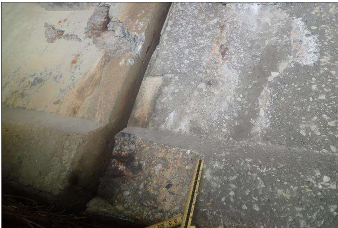
Span 2 Beam 3: (PAR) at bent 1, right face, spall/delamination (16 inch x full height x 2 inch deep) with exposed rusted strand
