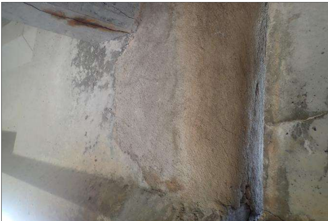
Span 2 Beam 1: PATCHED AREA FULL HEIGHT 1 FOOT LONG THAT IS SOUND ON RIGHT SIDE OVER PIER 2.
