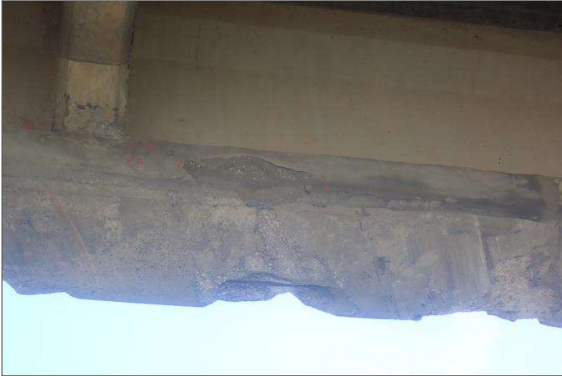
Span 3 Beam 4: (PAR) IMPACT - LEFT SIDE OF GIRDER LOCATED 18 FEET 2 INCHES FROM BENT 3- AREA OF PREVIOUS REPAIR DAMAGED - 1.417 FEET LONG X 7 INCHES HIGH X 1 INCH DEEP
