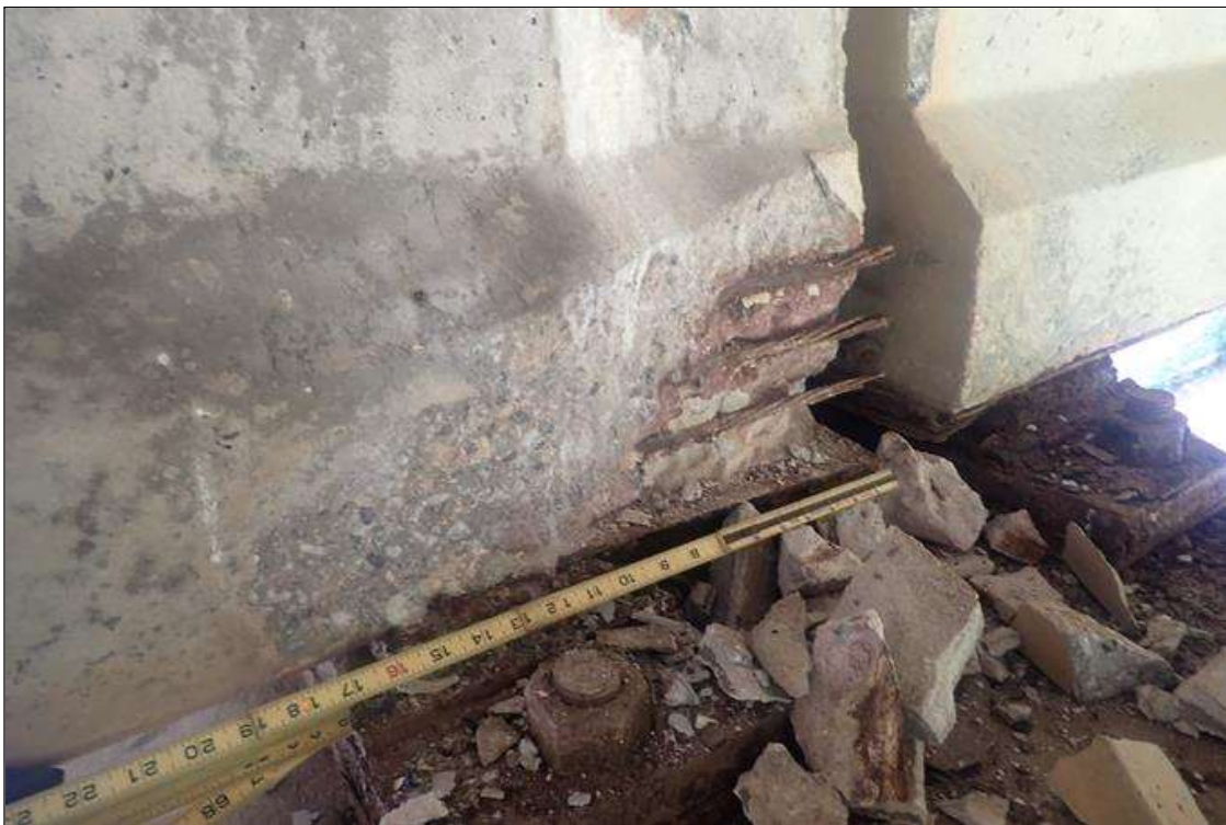
Span 3 Beam 3: (PAR) at bent 3, right face, bottom flange, failed patch (18 inch x 9 inch x 3 inch deep) with exposed rusted strands
