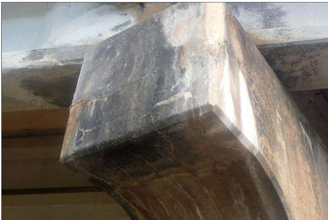
Bent 3 Cap 1: (PAR) both ends of cap, map cracks (hairline) with efflorescence buildup
