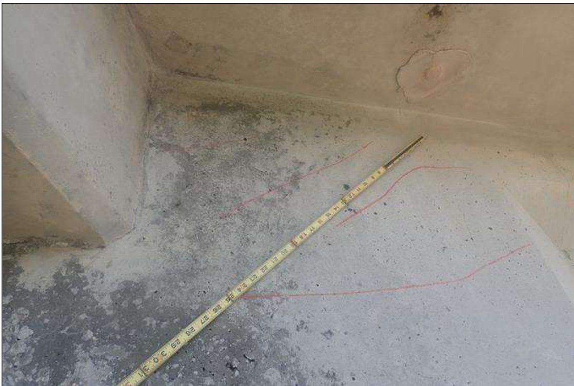
Span 3 Beam 1: 2 feet from bent 3, left face, top of web, multiple diagonal cracks (up to 0.008 inch x 4 feet)
