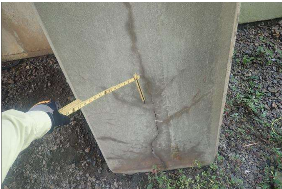
Bent 1 Pile 2: 1/8 inch vertical crack 3 feet long starting at ground line on south face, with map cracks (hairline)
