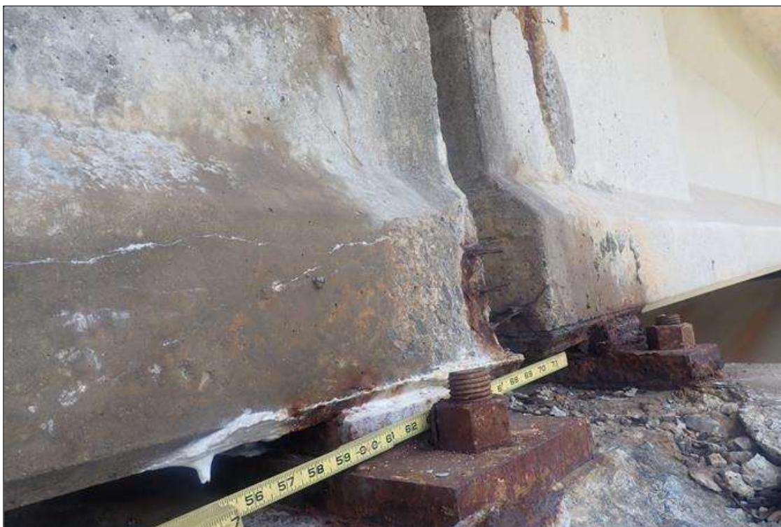
Span 2 Beam 1: (PAR) at bent 1, bottom flange, left side, spall (1 foot long x 8 inch high x 2 inch deep) with exposed rusted strand, and longitudinal cracks (up to 0.02 inch x 5 feet) with efflorescence buildup
