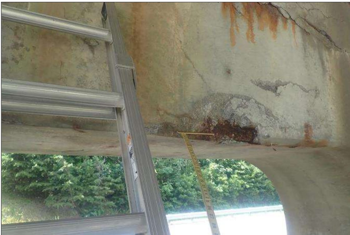
Bent 2 Cap 1: (PAR) south face, below bay 2, bottom corner, longitudinal crack (1/16 inch x 9.5 feet) with rust stains, and spall/delamination (3 feet x 1 foot x 2 inch deep) with exposed rusted rebar
