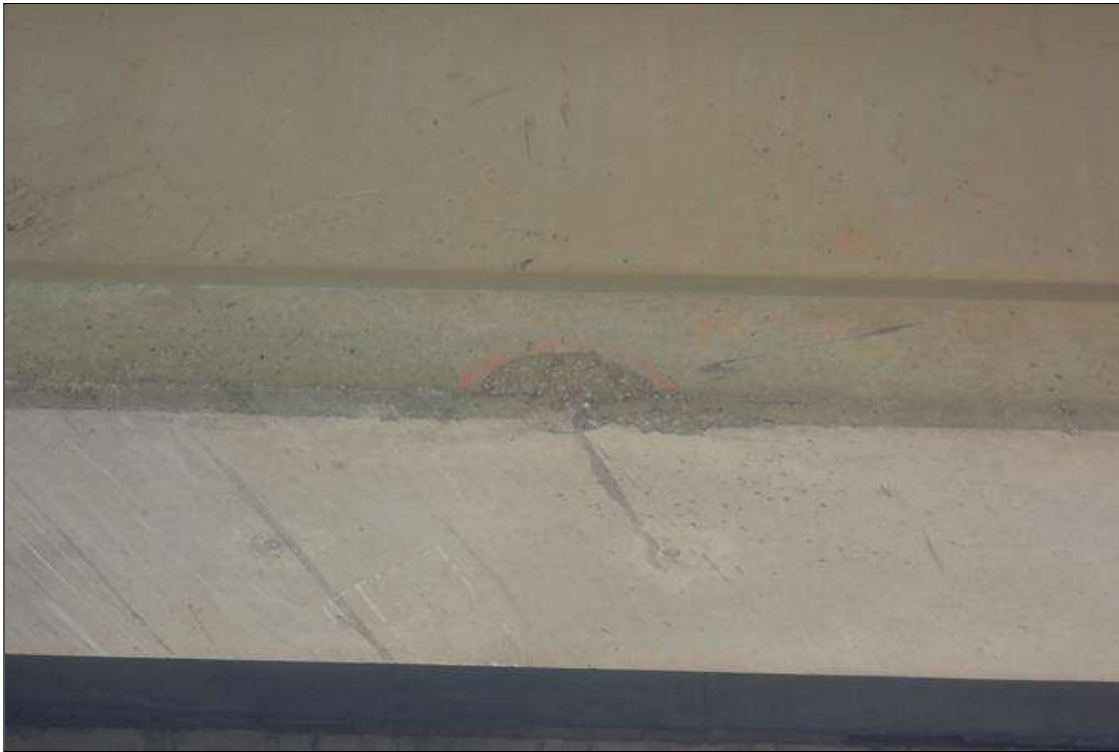
Span 3 Beam 3: (PAR) CHIPPED AREA FROM IMPACT DAMAGE ALONG BOTTOM EDGE OVER RIGHT LANE AND SEVERAL AREAS 3 INCHES X 5 INCHES - 02/16/2023 - IMPACT DAMAGE - LOCATED 11 FEET 2 INCHES FROM BENT 3; AREA DIMENSIONS ARE 10 INCHES LONG X 4 INCHES WIDE X 1/2 INCH DEEP ON NORTH SIDE OF BOTTOM FLANGE - 07/07/2023 no apparent change since supplemental inspection
