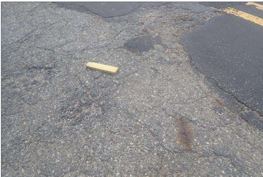
Span 2 Wearing Surface: SEVERAL AREAS TRANSVERSE AND MAP CRACKING / DETERIORATED ASPHALT WITH CRACKS UP TO 1/2 INCH, SOME WITH RUST STAINS, SOME AREAS DELAMINATED
