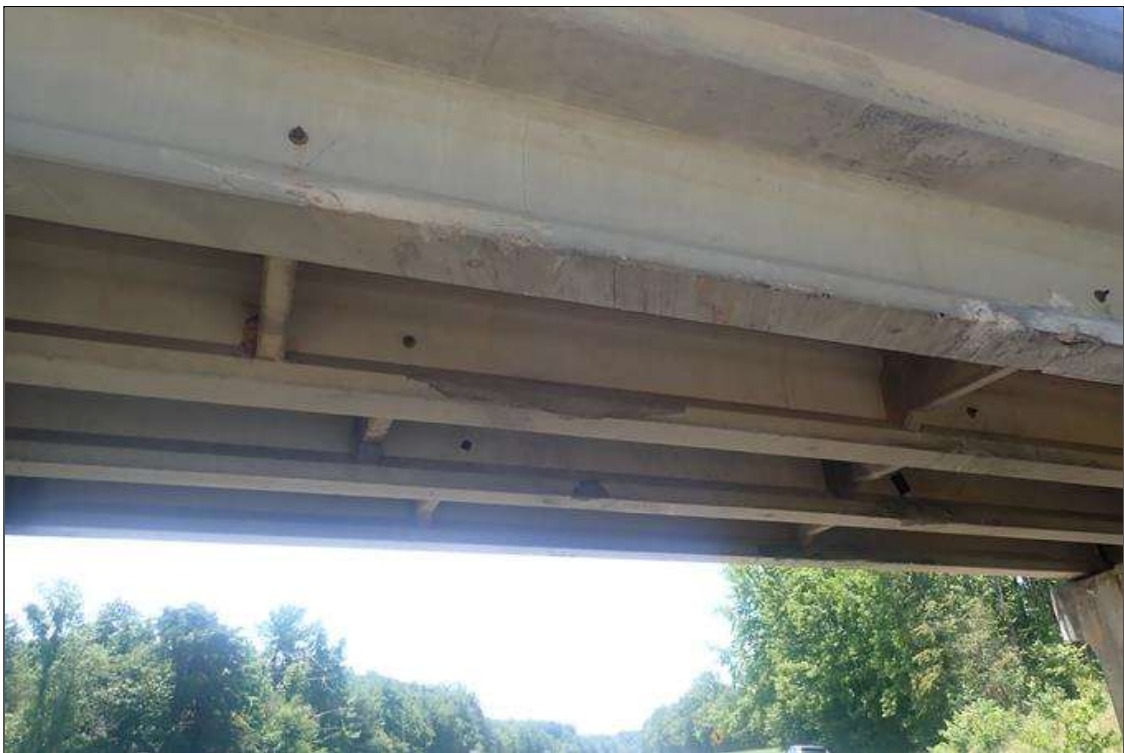
span 3, beam 4, impact damage over left southbound lane, overview
