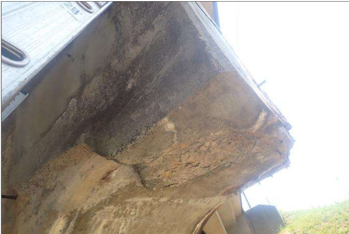
Bent 1 Cap 1: (PAR) west end of cap, delaminated/partially failed previous repair (3.5 feet long x full height x full width), with spalls (up to 2 feet x 16 inch x 2 inch deep) with exposed rusted rebar, rust stains, efflorescence buildup, and cracks (up to 1/8 inch)
