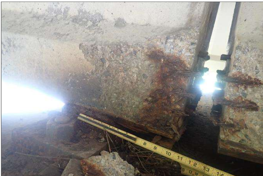
Span 2 Beam 3: (PAR) 8 INCH LONG X 1 FOOT HIGH X 2 INCH DEEP spall with exposed strands on right bottom flange at pier 2
