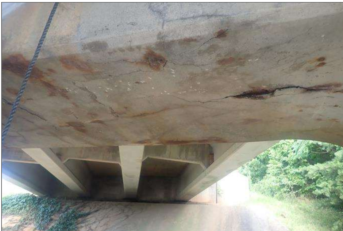
Bent 3 Cap 1: (PAR) underside, between columns, delamination/spall (18 feet x full width x 1 inch deep) with exposed rusted rebar, with cracks (up to 1/16 inch) and rust stains
