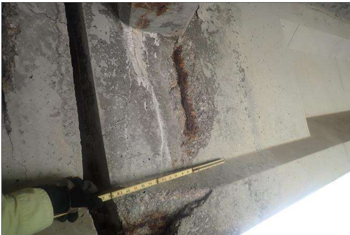
Span 2 Beam 3: (PAR) at bent 2, web, left face, delamination/spall (20 inch x 24 inch x 1 inch deep) with exposed rusted rebar, with cracks (0.02 inch) extending onto right face, and efflorescence buildup
