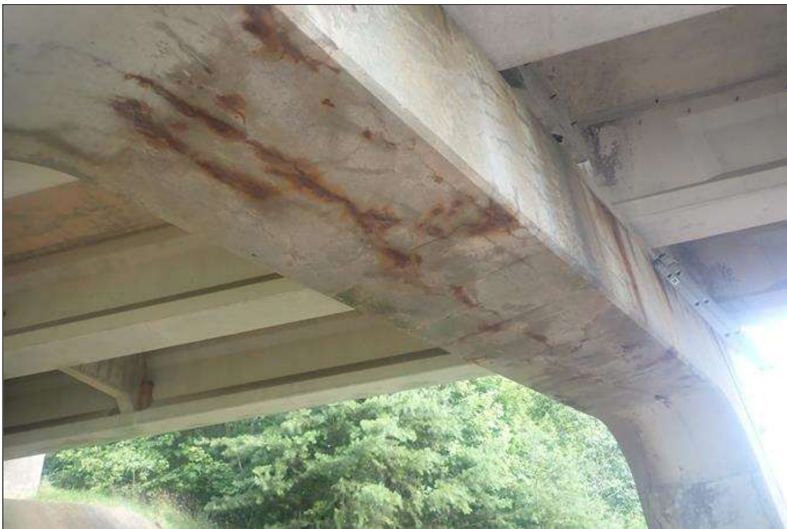
Bent 3 Cap 1: (PAR) underside, between columns, delamination/spall (18 feet x full width x 1 inch deep) with exposed rusted rebar, with cracks (up to 1/16 inch) and rust stains
