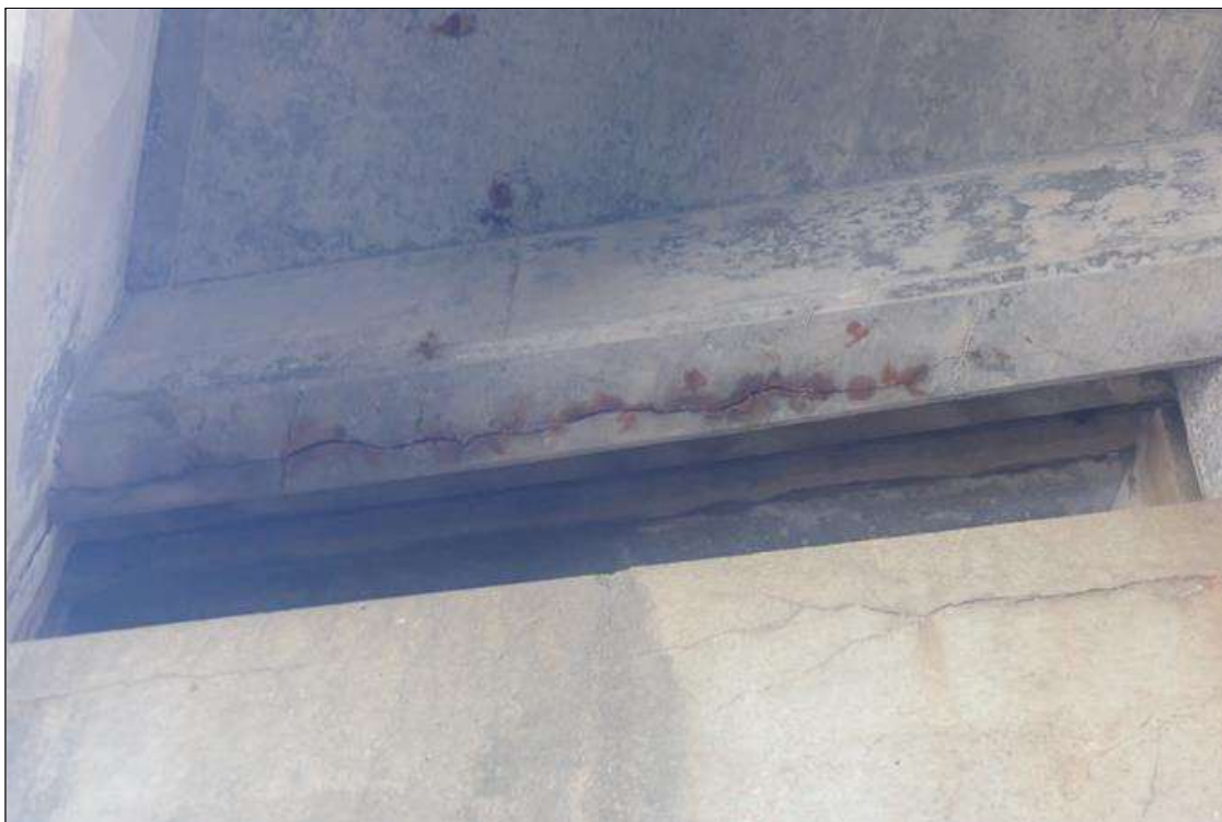
Span 2 Deck: (PAR) bent 1 end diaphragm, bays 1, 2, 3 and right overhang, longitudinal cracks (up to 1/8 inch x 6 feet long) with rust stains and some efflorescence buildup
