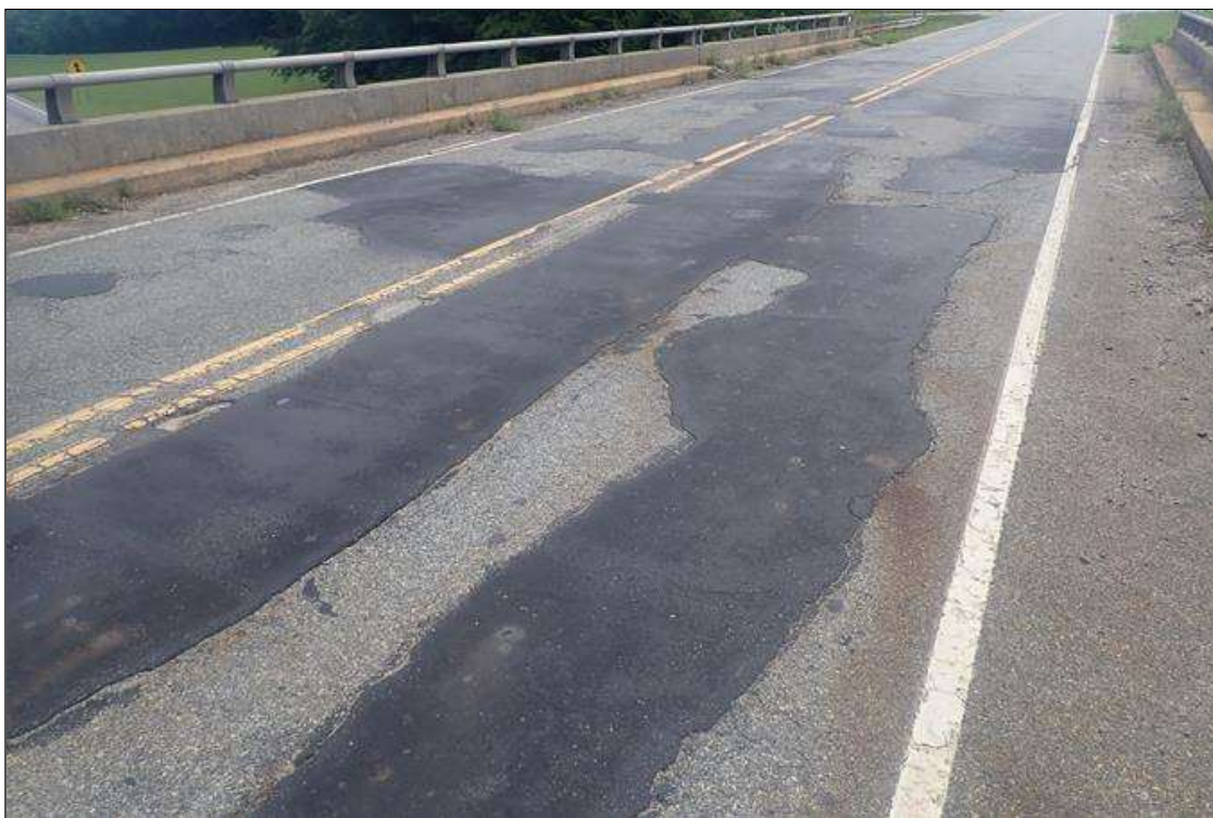
Span 2 Wearing Surface: Several large sound asphalt patches in travel lanes
