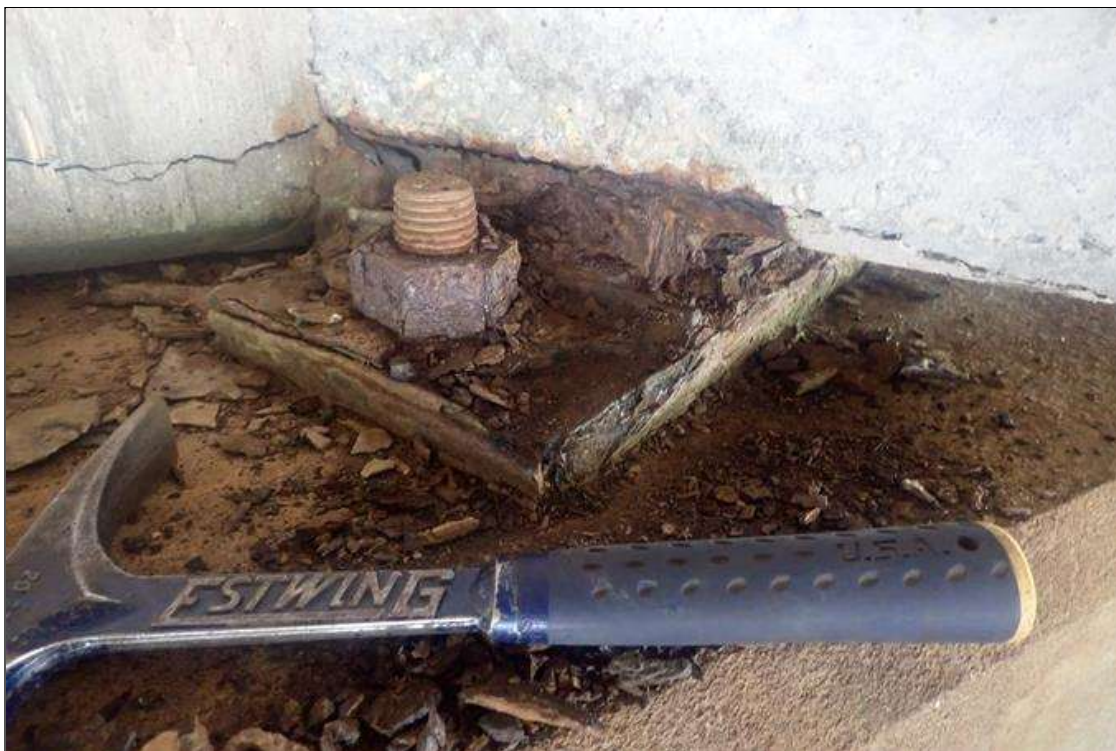
Span 4 Beam 4 - Far Bearing 4: rust scale/pack rust
