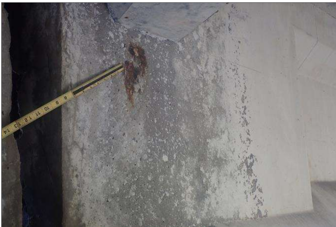
Span 1 Beam 4: (PAR) at bent 1, left face, web, rust stains (3 inch)
