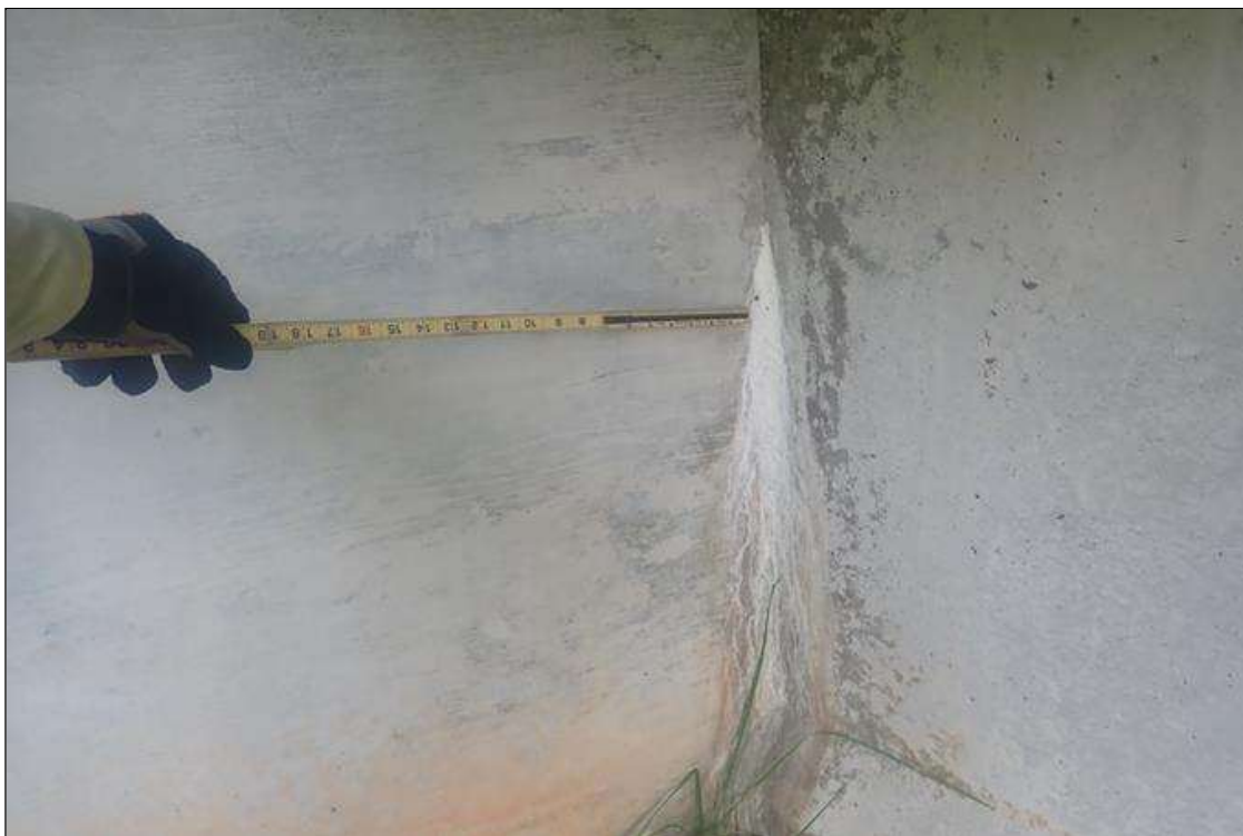
End Bent 1 Abutment: (PAR) right end, at beam 4 web, efflorescence buildup
