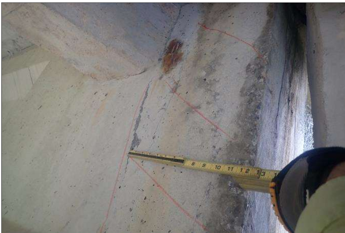
Span 1 Beam 1: (PAR) at bent 1, web, right face, delamination (12 inch x full height) with rust stains; end face, (2) vertical cracks (0.06 inch x full height)
