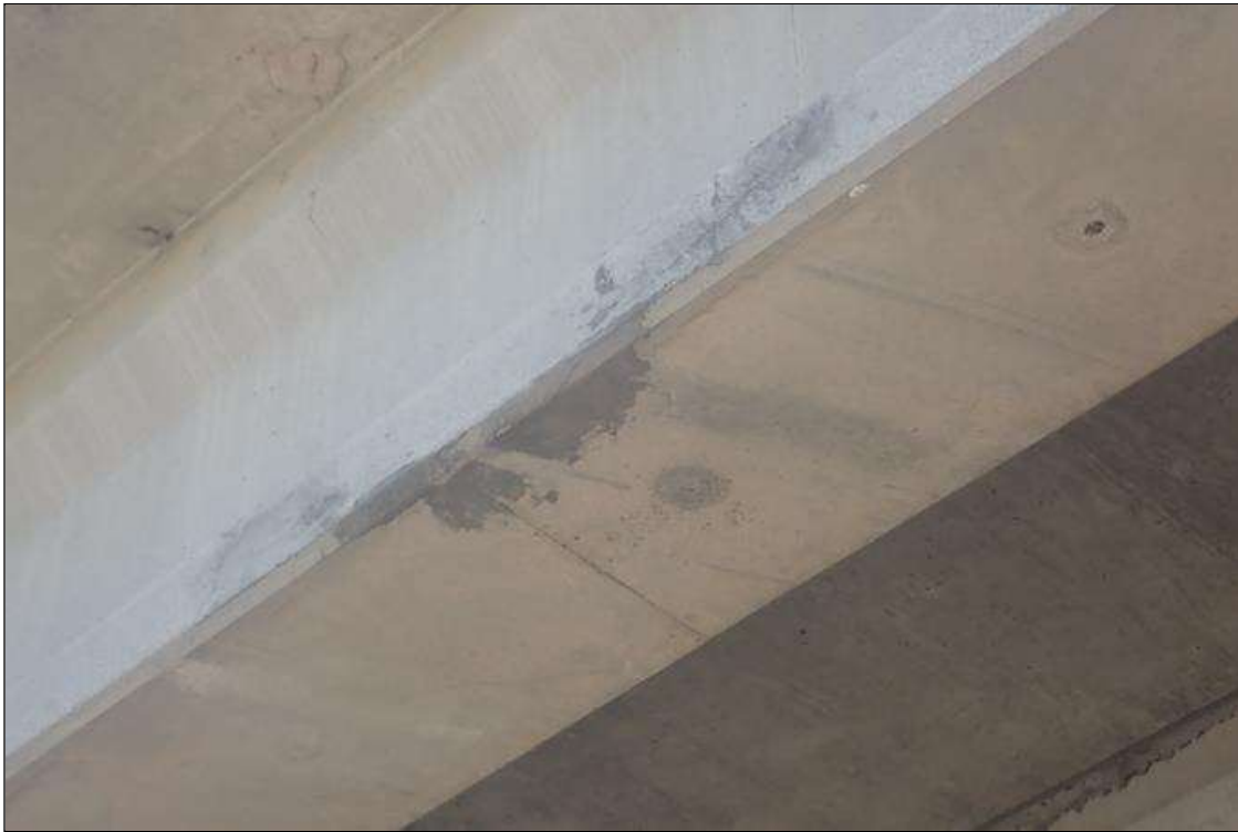
Span 3 Beam 1: 10 feet north of 1st intermediate diaphragm, bottom flange, left corner, patch (approximately 2 feet x 6 inch)
