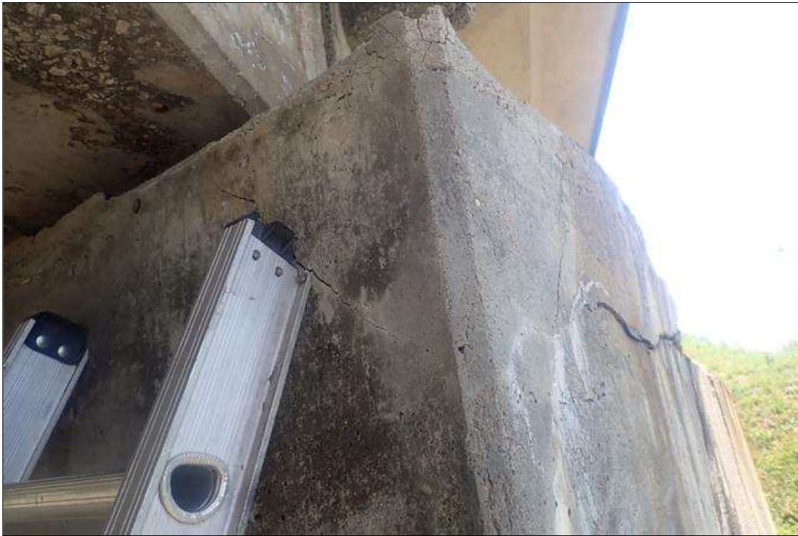
Bent 1 Cap 1: (PAR) west end of cap, delaminated/partially failed previous repair (3.5 feet long x full height x full width), with spalls (up to 2 feet x 16 inch x 2 inch deep) with exposed rusted rebar, rust stains, efflorescence buildup, and cracks (up to 1/8 inch)
