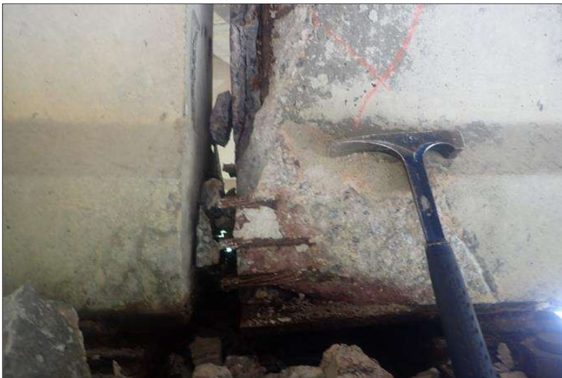
Span 3 Beam 3: (PAR) at bent 3, left face, failed patch/spall (12 inch x 39 inch x 3 inch deep) with exposed rusted strands and rebar, with efflorescence buildup at diaphragm
