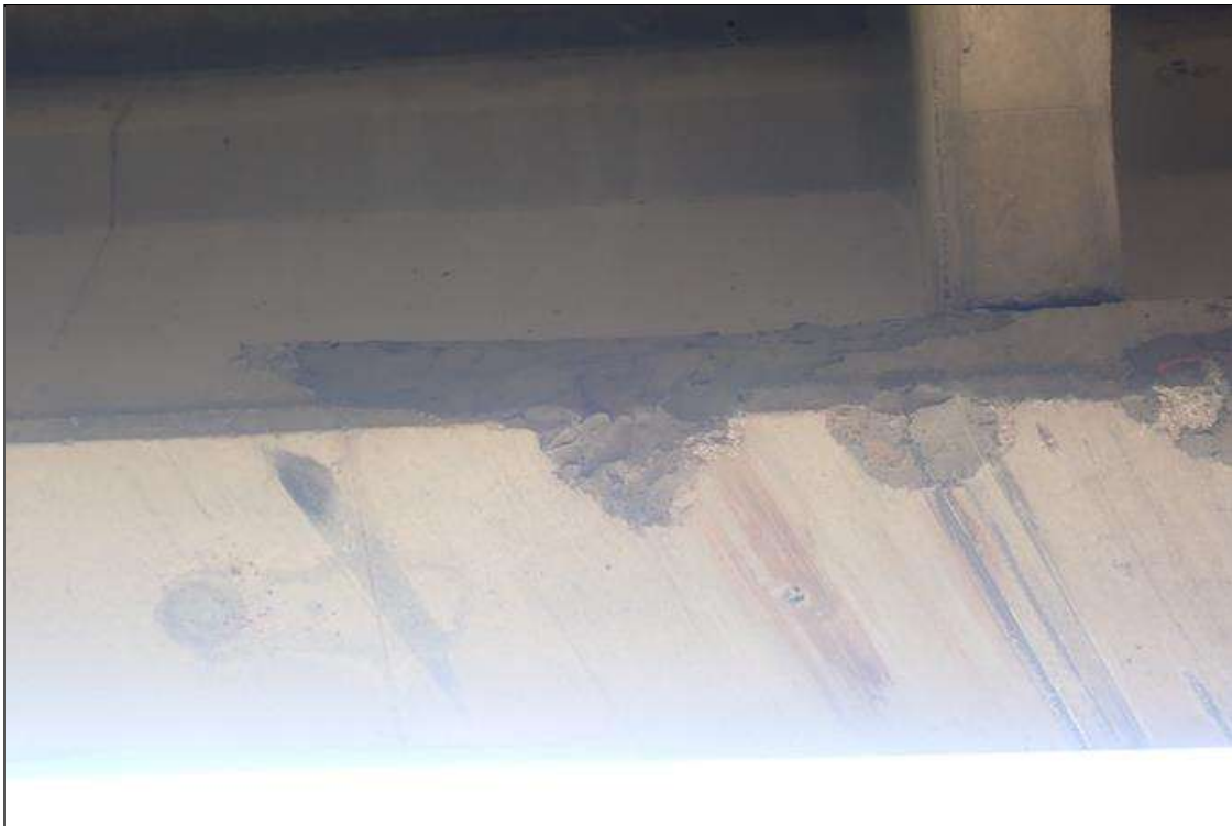
Span 3 Beam 1: (PAR) south side of second intermediate diaphragm, bottom flange, right face, patch (approximately 2 feet x 8 inch) with map cracks (approximately 1/32 inch), potentially delaminated
