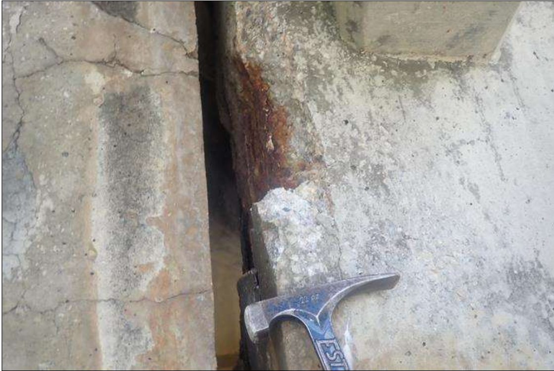
Span 2 Beam 4: (PAR) at bent 1, end of web, spall/delamination (30 inch high x full width x 2 inch deep) with exposed rusted rebar (up to 1/8 inch loss), extends along face of web (up to 10 inch)
