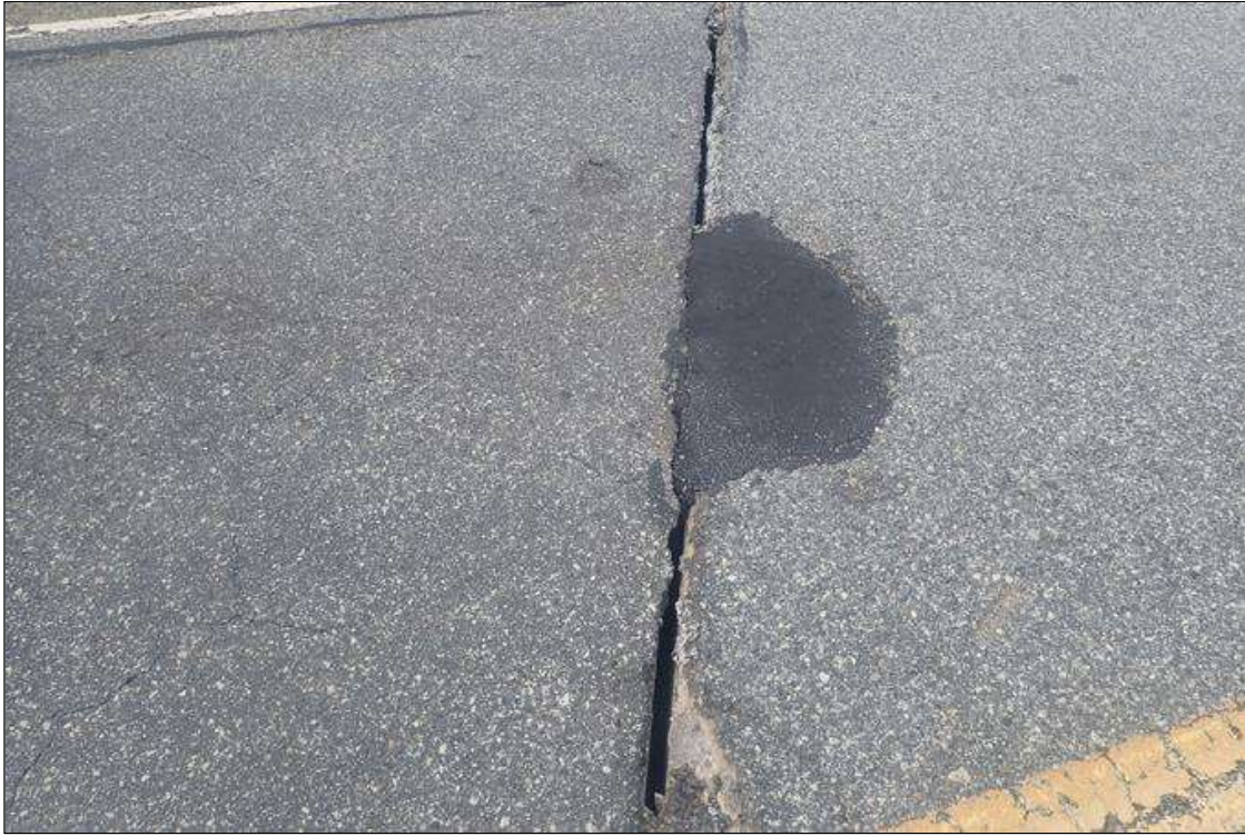
Span 3 Wearing Surface: ASPHALT PATCH MISSING OVER PIER 3 JOINT 9 FEET LONG. JOINT IS MISSING WITH TOP OF CAP VISIBLE THROUGH OPENING.
