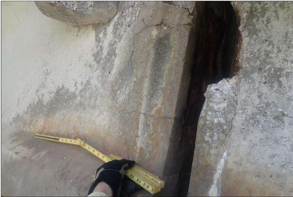
Span 1 Beam 4: (PAR) at bent 1, end of web, spall (30 inch high x 10 inch wide x 1 inch deep) with exposed rusted rebar, with delamination extending along right face with map cracks (up to 0.03 inch x 2 feet x full height)
