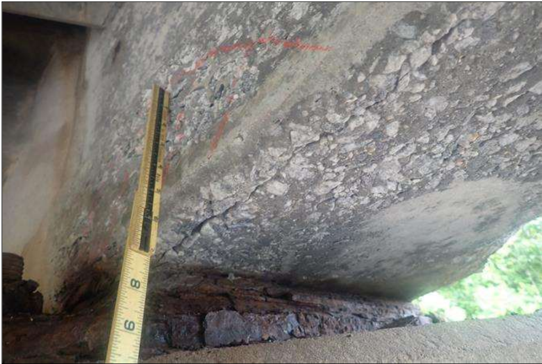
Span 3 Beam 4: (PAR) at bent 3, left face, bottom flange, delamination (12 inch x 6 inch) with (2) longitudinal cracks (up to 1/16 inch x 2 feet)
