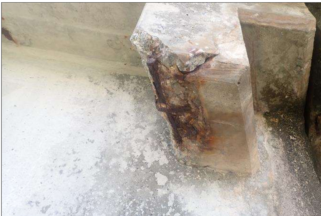
Span 3 Deck: bent 2 end diaphragm, left overhang, spall (12 inch x 6 inch x 2 inch deep) with exposed rusted rebar
