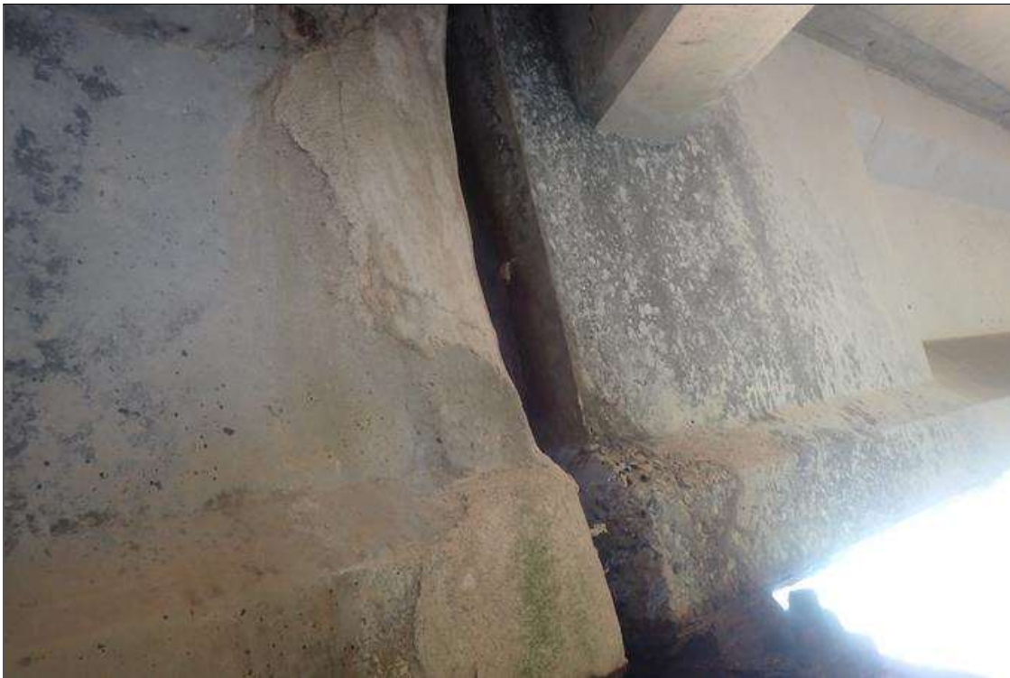
Span 3 Beam 1: FULL HEIGHT PATCHED AREA BOTTOM FLANGE AND WEB 10 INCHES LONG THAT IS SOUND ON RIGHT SIDE OVER PIER 3.
