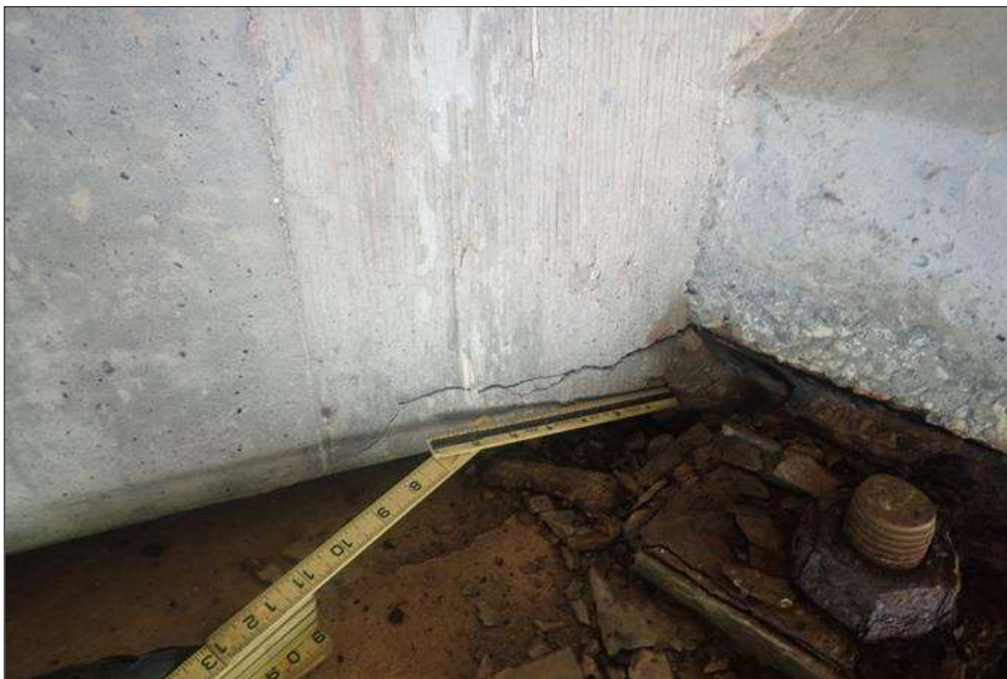
End Bent 2 Abutment: at multiple bottom flanges, longitudinal crack (up to 1/16 inch x 12 inch)
