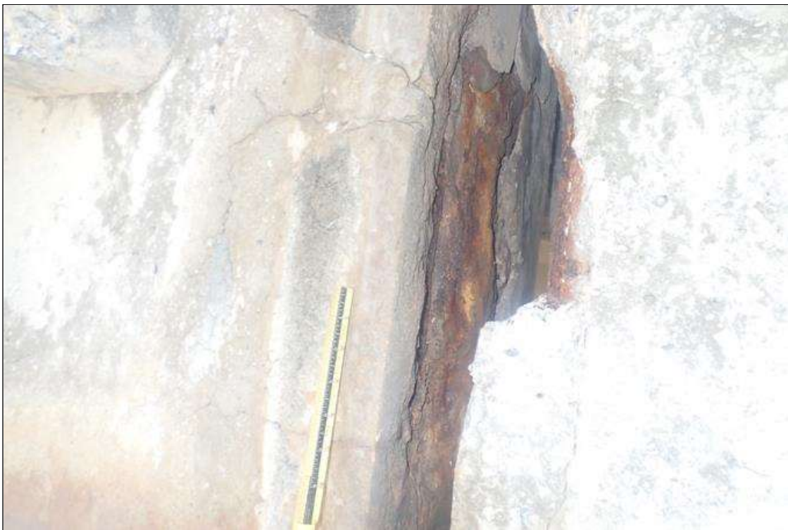
Span 1 Beam 4: (PAR) at bent 1, end of web, spall (30 inch high x 10 inch wide x 1 inch deep) with exposed rusted rebar, with delamination extending along right face with map cracks (up to 0.03 inch x 2 feet x full height)
