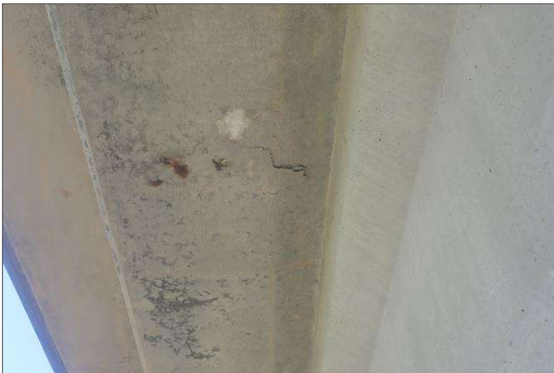
Span 2 Deck: (PAR) left overhang, 4 feet from bent 1, delamination (2 feet x 5 inch) with rust stains
