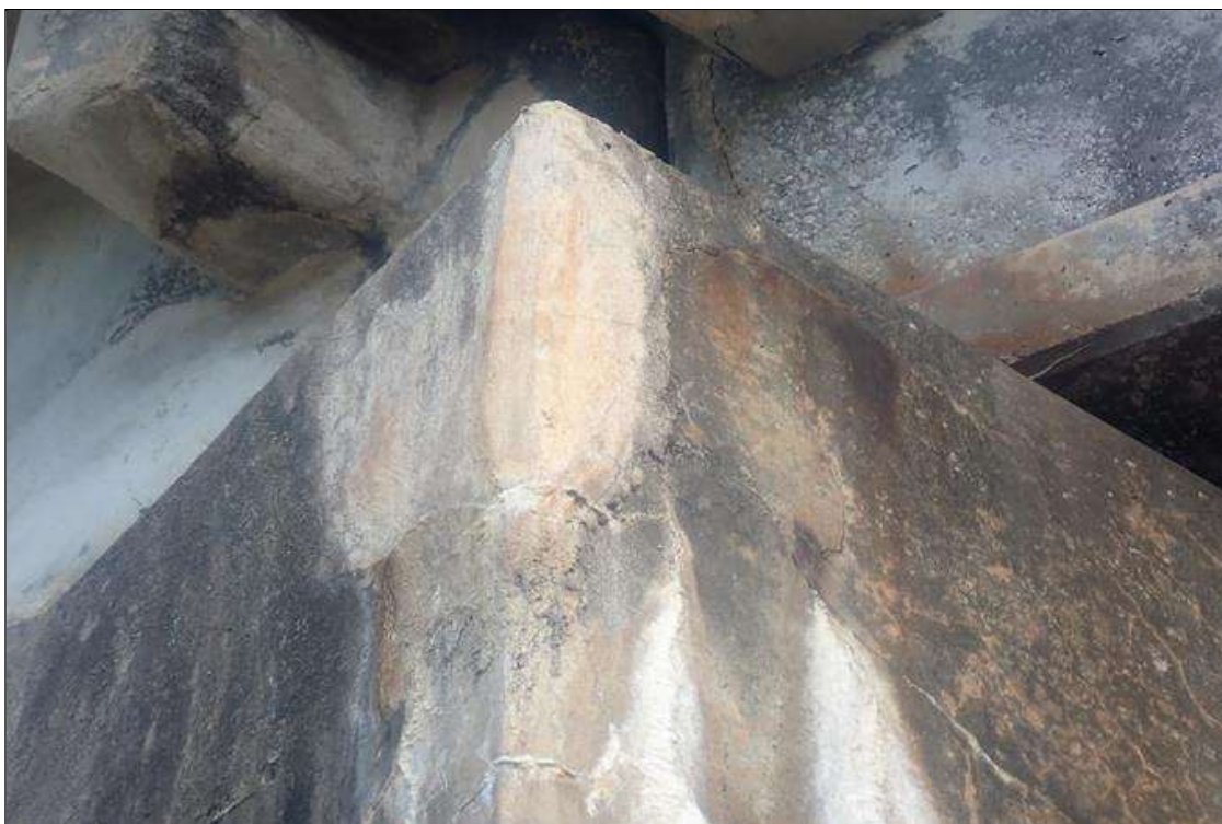
Bent 3 Cap 1: southwest corner, at top, patch (6 inch x 12 inch)
