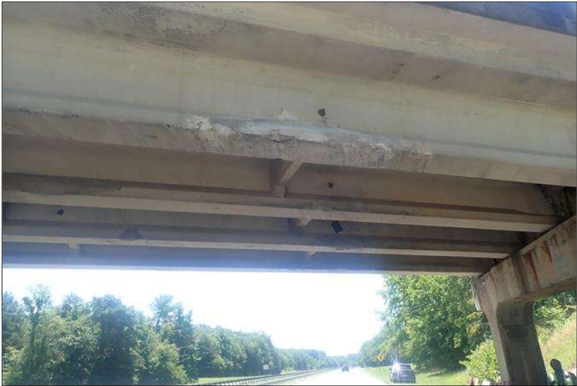
span 3, beam 4, impact damage over right southbound lane, overview
