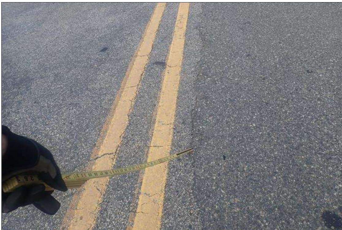
Span 3 Wearing Surface: FULL LENGTH 1/2 INCH LONGITUDINAL CRACK NEAR CENTERLINE
