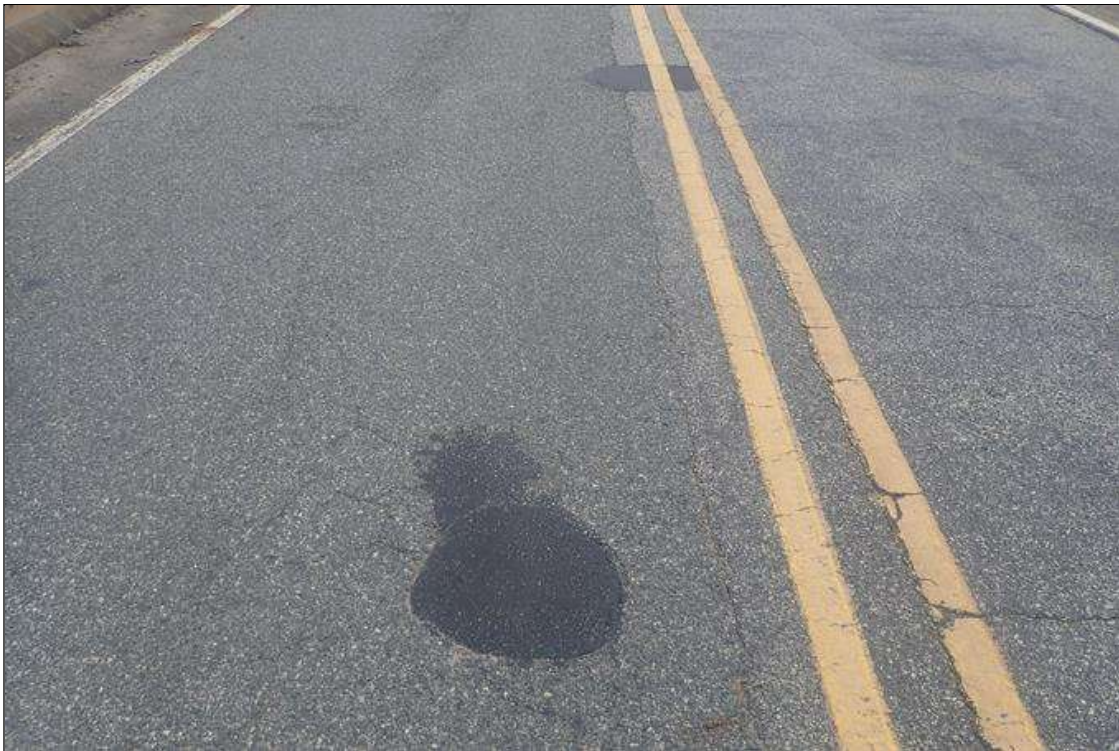
Span 3 Wearing Surface: TWO SOUND ASPHALT PATCHED AREAS UP TO 2 FEET X 2 FEET IN NORTH BOUND TRAVEL LANE
