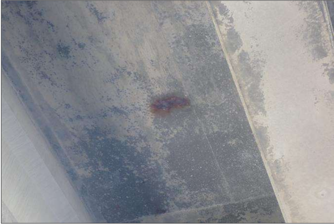
Span 2 Deck: (PAR) underside, at random, areas of transverse/map cracks (hairline) with rust stains
