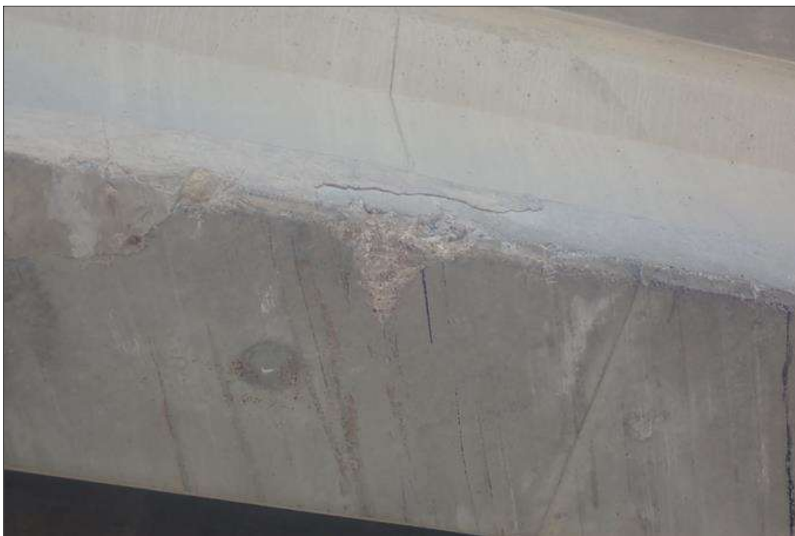
Span 3 Beam 4: (PAR) 25 feet from bent 2, over left southbound lane, bottom flange, right face, impact spall (approximately 10 inch x 6 inch x 2 inch deep)
