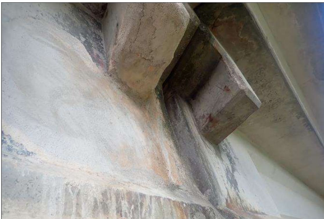
Span 3 Beam 4: FULL HEIGHT X UP TO 3 FEET LONG PATCHED AREA THAT IS SOUND ON WEB AND BOTTOM FLANGE BOTH SIDES OVER PIER 3.
