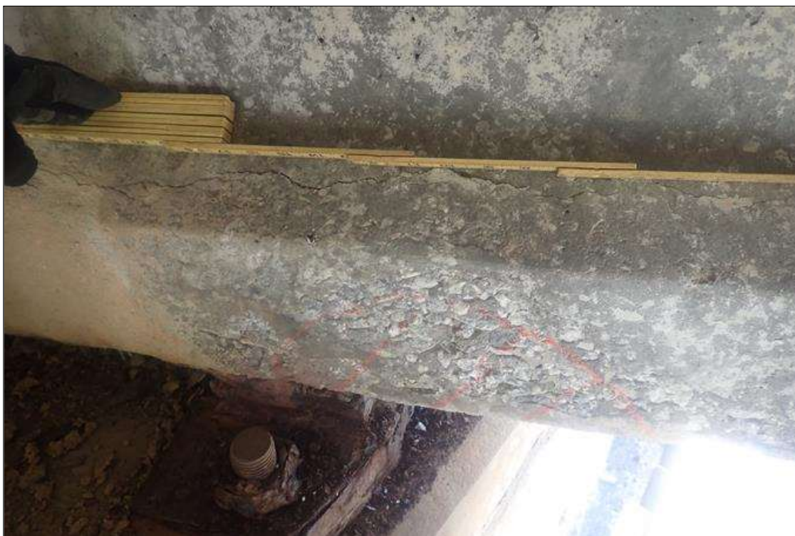
Span 3 Beam 4: (PAR) at bent 3, left face, bottom flange, delamination (12 inch x 6 inch) with (2) longitudinal cracks (up to 1/16 inch x 2 feet)
