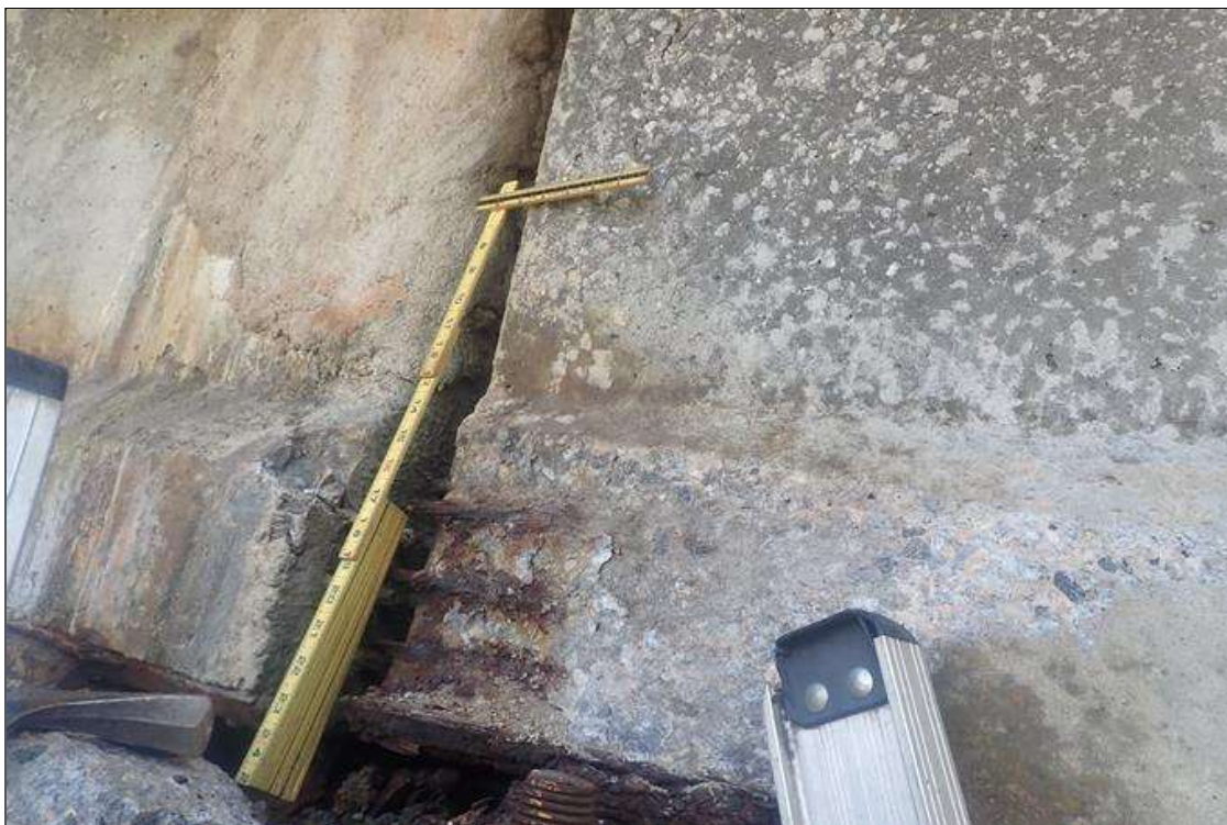
Span 3 Beam 4: (PAR) at bent 2, bottom flange, right face, spall (16 inch x 8 inch x 2 inch deep) with exposed rusted strands; web, delamination (4 inch x full height)
