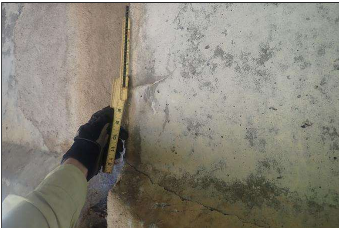
Span 3 Beam 1: at bent 2, right face, web, map cracks (hairline x 6 inch x 8 inch) with efflorescence
