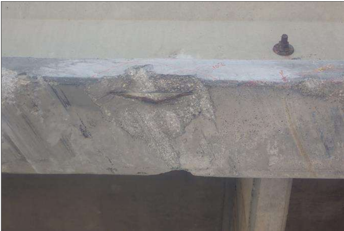
Span 3 Beam 4: (PAR) 5 FEET LONG PATCHED AREA THAT IS SOUND ON ALONG EAST SIDE OF BOTTOM FLANGE OVER LEFT SOUTHBOUND TRAVEL LANE - 02/16/2023 - IMPACT - LOCATED 18 FEET 2 INCHES FROM BENT 3 - DIMENSIONS ARE 10 INCHES LONG X 1.583 FEET WIDE X 4 INCHES DEEP; WITH EXPOSED TENSION CABLE - 07/07/2023 no apparent change from supplemental inspection
