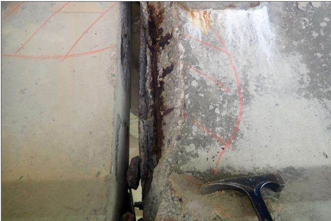
Span 3 Beam 3: (PAR) at bent 3, left face, failed patch/spall (12 inch x 39 inch x 3 inch deep) with exposed rusted strands and rebar, with efflorescence buildup at diaphragm
