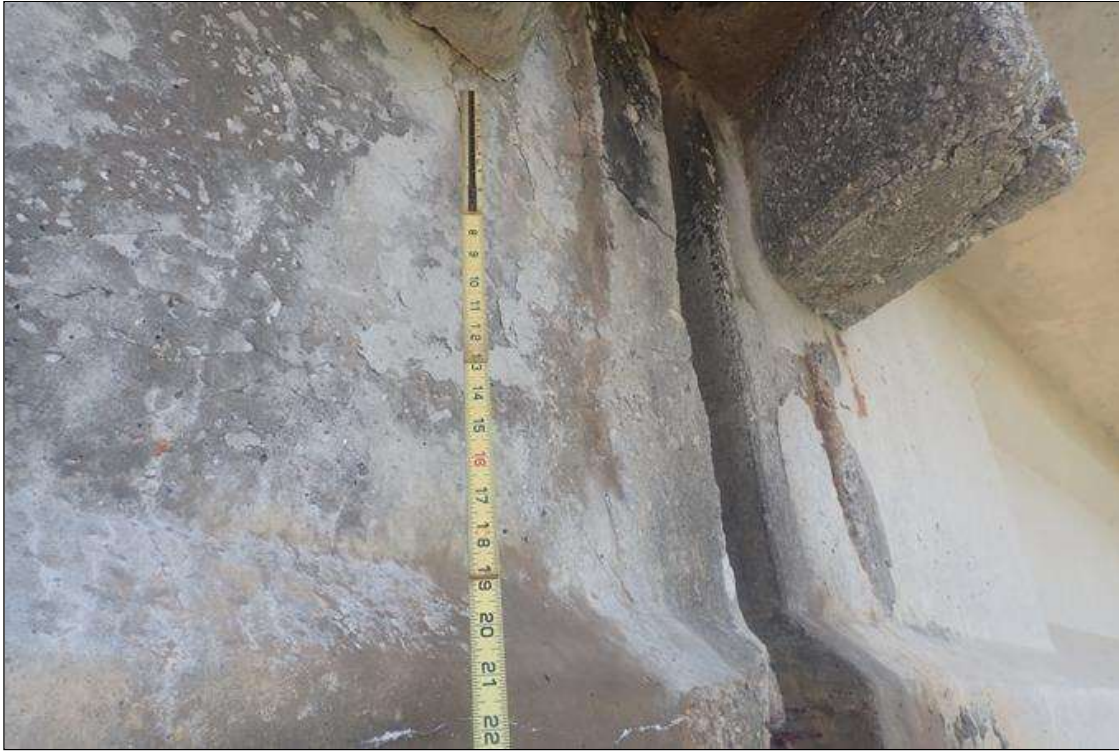
Span 2 Beam 1: 12 INCH WIDE X FULL HEIGHT DELAMINATION IN LEFT SIDE WEB AT BENT 1
