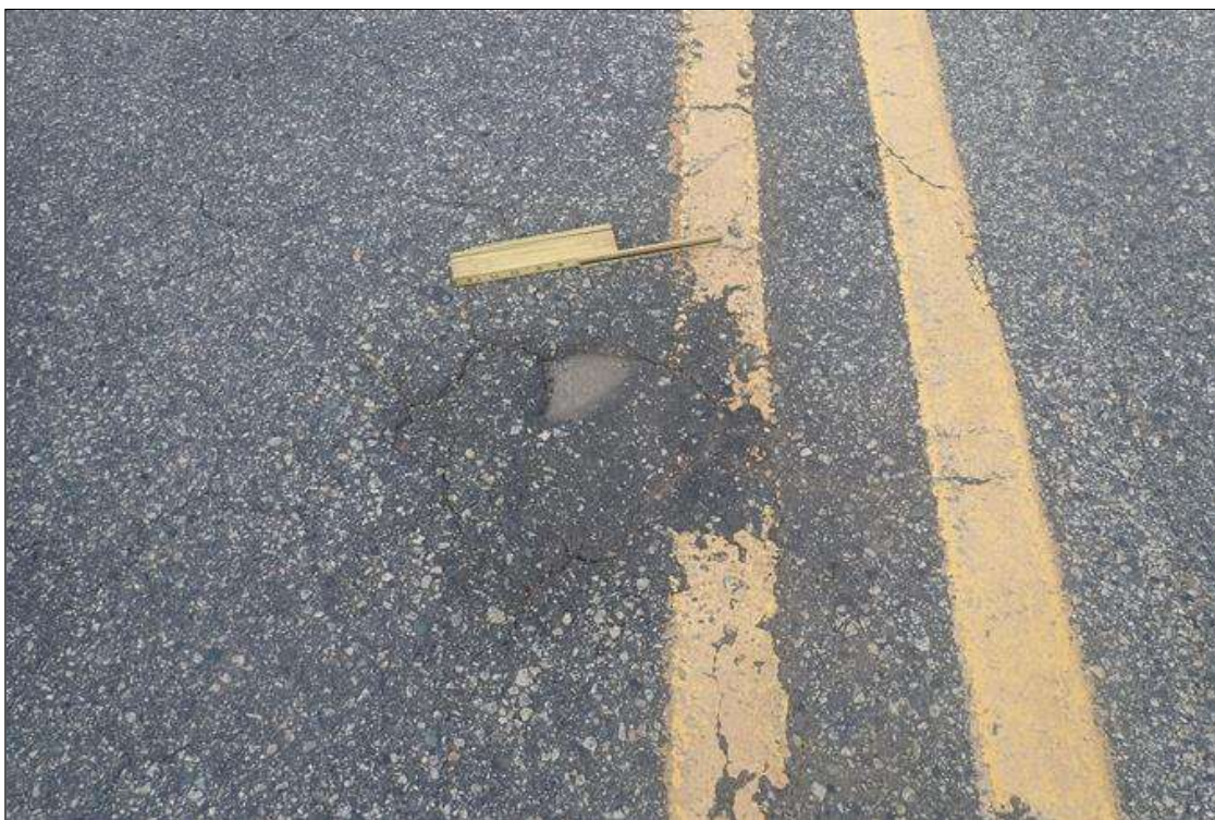
Span 3 Wearing Surface: centerline, near bent 3, (2) potholes (up to 12 inch diameter x full depth)
