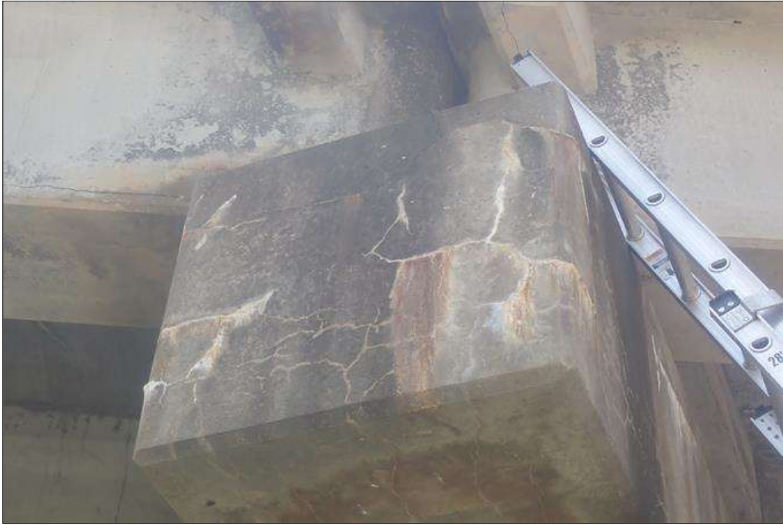
Bent 2 Cap 1: (PAR) hairline to 1/32 inch map cracking with efflorescence buildup and rust stains on west face cap
