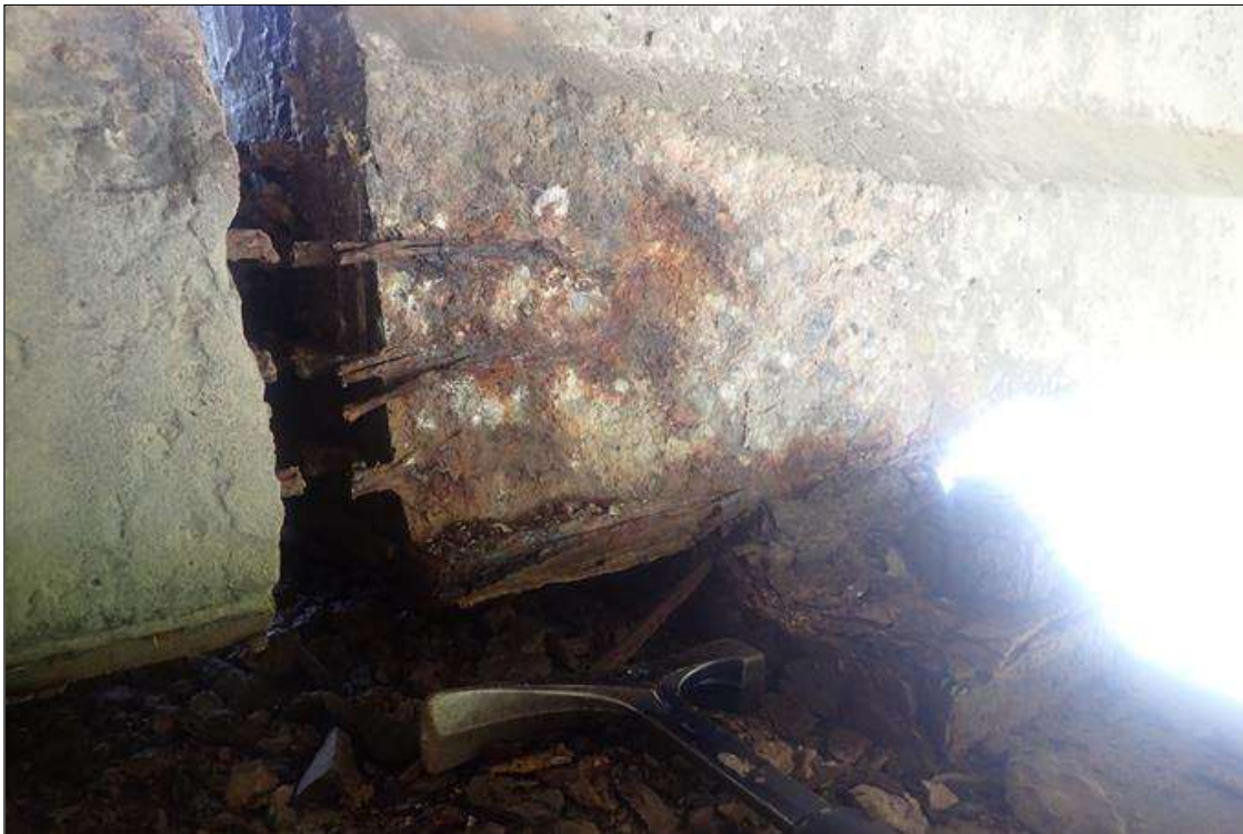
Span 2 Beam 4: (PAR) 9 INCH HIGH X 1 FOOT LONG X 2 INCH DEEP SPALL ON LEFT SIDE BOTTOM FLANGE WITH 3 STRANDS EXPOSED WITH 1/16 INCH SECTION LOSS OVER PIER 2.
