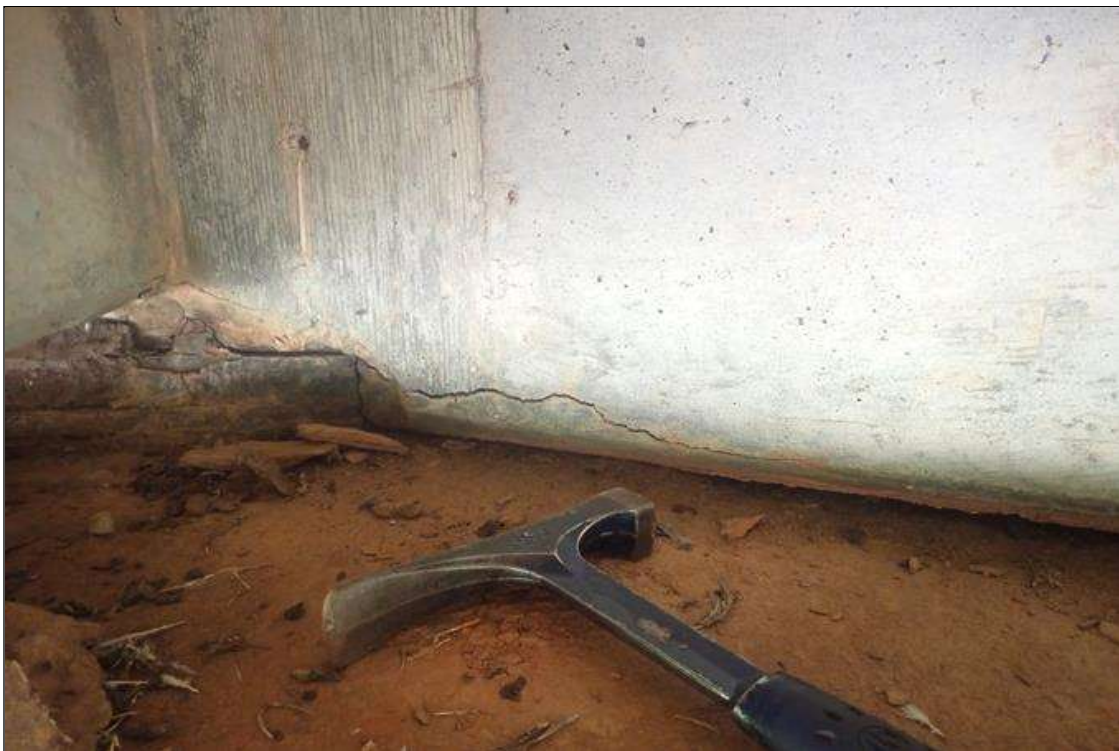
End Bent 1 Abutment: 1/16 inch horizontal cracks up to 1 foot long, some with efflorescence, starting at bottom corner of beams all bays
