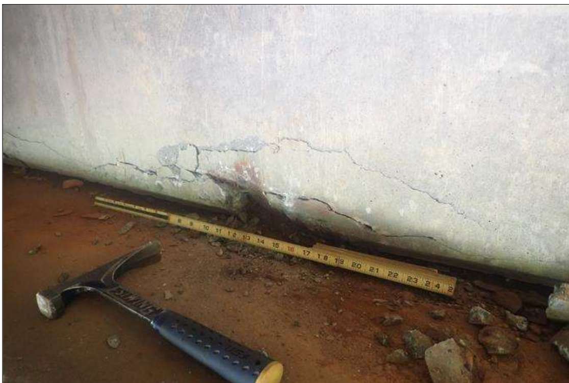
End Bent 2 Abutment: bay 2, bottom corner, spall/delamination (2 feet x 6 inch x 2 inch deep) with exposed rusted rebar
