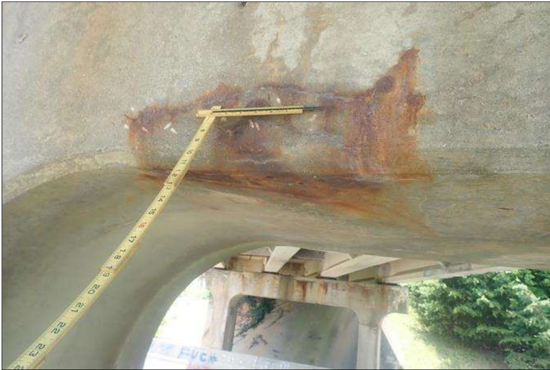
Bent 2 Cap 1: (PAR) south face blow bay 1, bottom corner, longitudinal crack (1/32 inch x 2 feet) with rust stains
