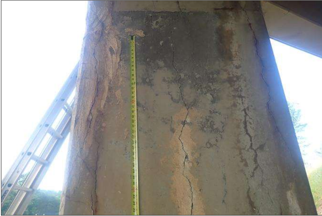
Bent 3 Pile 1: (PAR) VERTICAL CRACKING UP TO 1/8 INCH AND DELAMINATION UP TO 6 INCH WIDE ON ALL 4 SIDES WITH SOME OF CRACKS SEALED OVER BUT STILL CRACKED THROUGH TOP TO BOTTOM WITH RUST STAINS.
