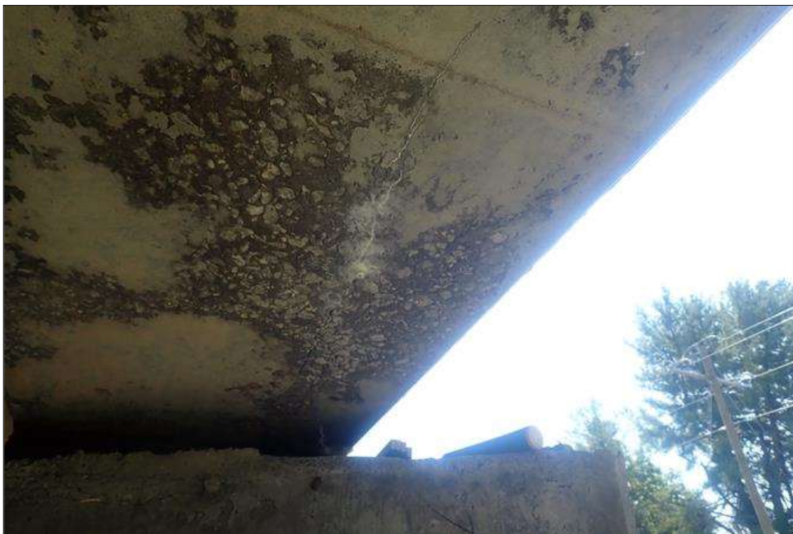
Span 2 Beam 1: (PAR) at bent 1, bottom flange, left side, spall (1 foot long x 8 inch high x 2 inch deep) with exposed rusted strand, and longitudinal cracks (up to 0.02 inch x 5 feet) with efflorescence buildup
