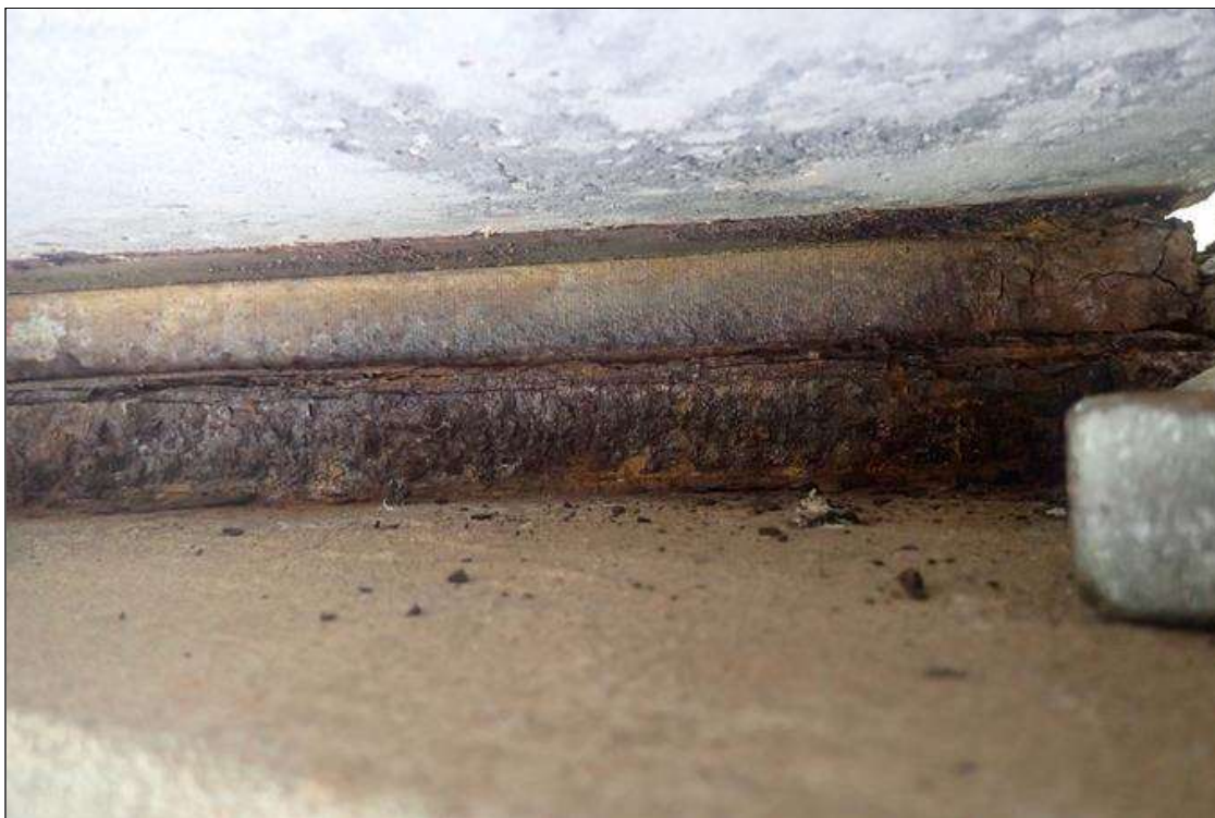
Span 2 Beam 2 - Near Bearing 2: rust scale/pack rust
