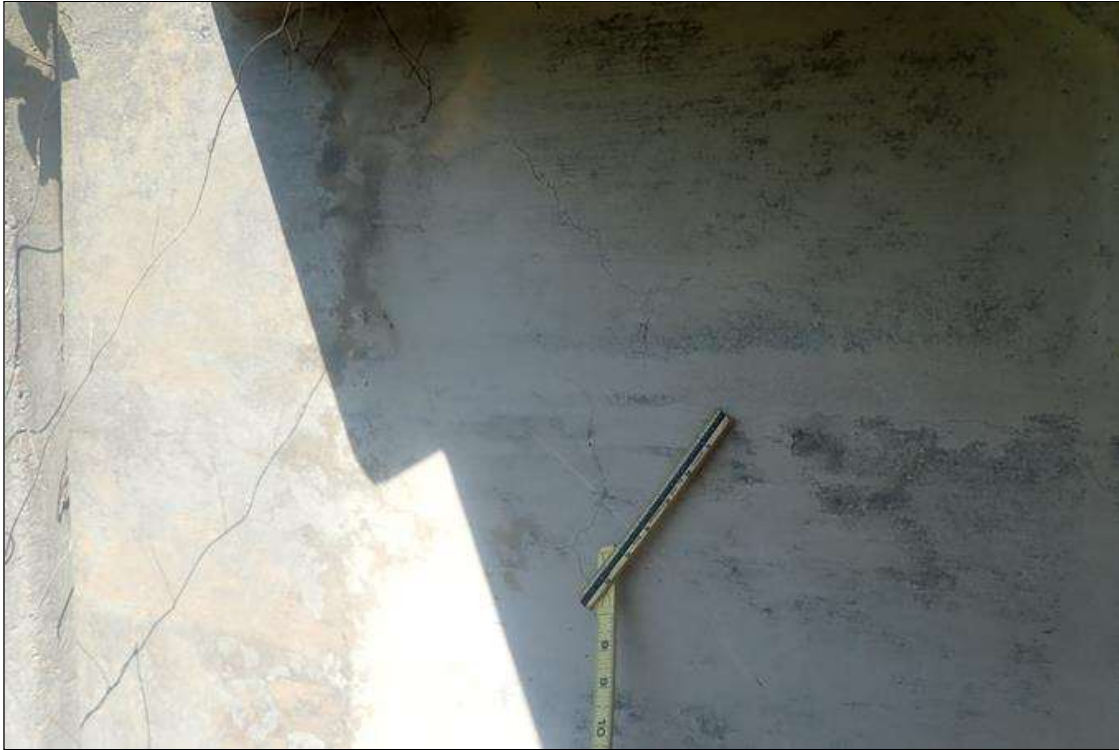
End Bent 2 Abutment: left end, map cracks (hairline x 2 feet x 2 feet)
