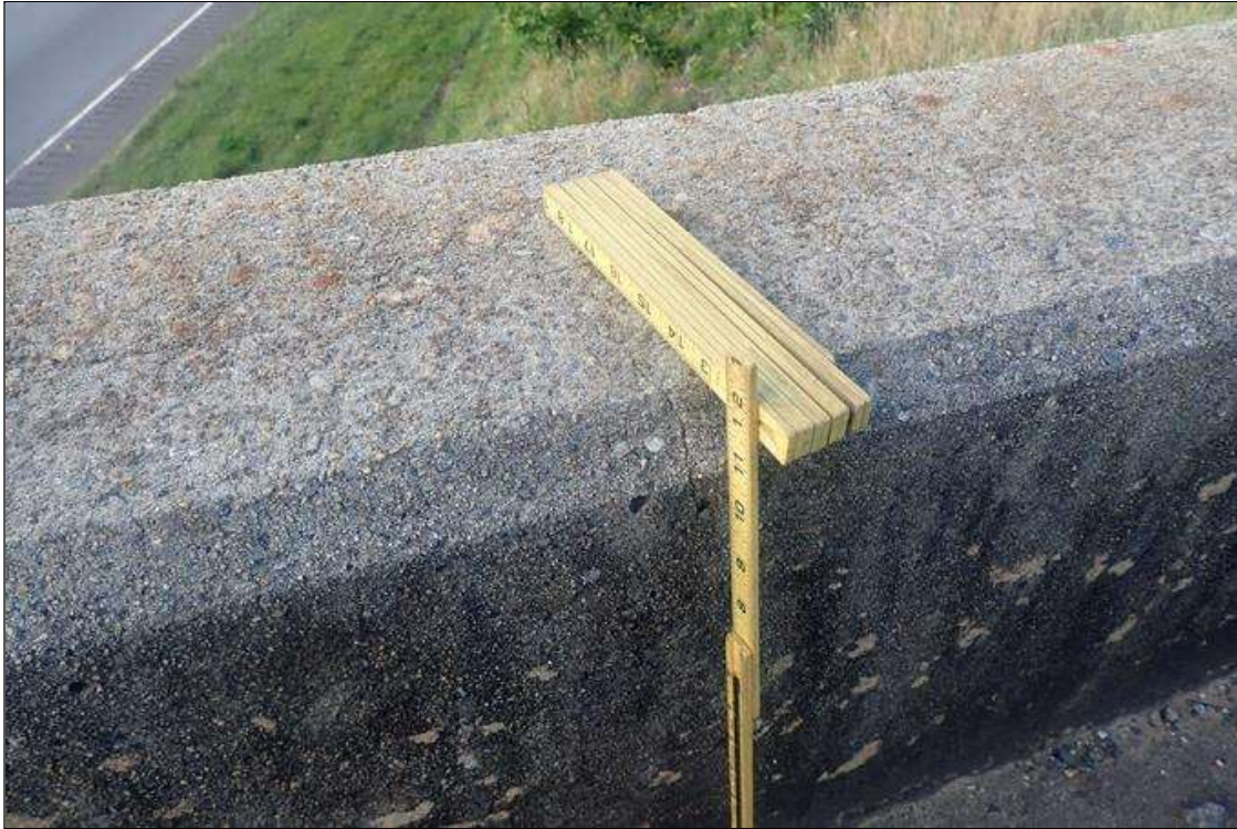
Span 4 Left Bridge Rail: HAIRLINE MAP CRACKING IN CURB PORTION OF RAIL AND HAIRLINE TRANSVERSE CRACKS IN TOP OF PARAPET AT VARIOUS LOCATIONS ALONG RAIL
