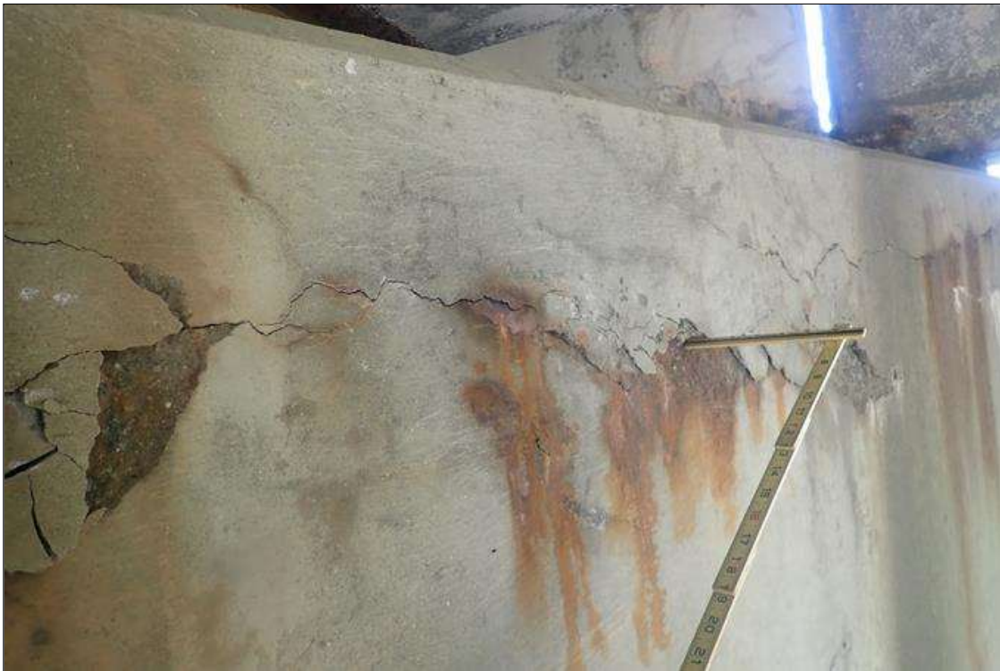
Bent 2 Cap 1: (PAR) HORIZONTAL CRACKING UP TO 1/4 INCH WITH DELAMINATIONS/SPALLS (UP TO 1 INCH DEEP), EFFLORESCENCE BUILDUP AND RUST STAINS AT TOP EDGE ALONG LENGTH OF BOTH FACES.
