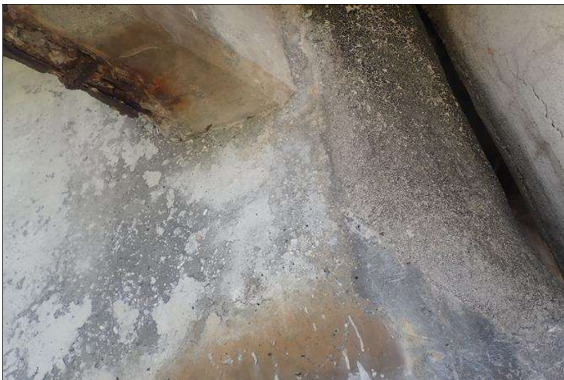
Span 3 Beam 1: 1 FOOT LONG SOUND PATCHED FULL HEIGHT OF WEB AT BEAM END, LEFT FACE AT PIER 2.
