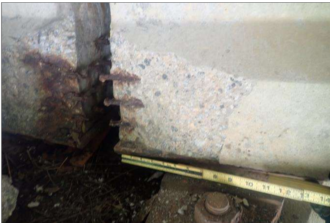
Span 3 Beam 3: (PAR) 8 INCHES LONG X 8 INCHES HIGH X 2 INCHES DEEP SPALL WITH EXPOSED STRANDS ON RIGHT BOTTOM FLANGE AT PIER 2
