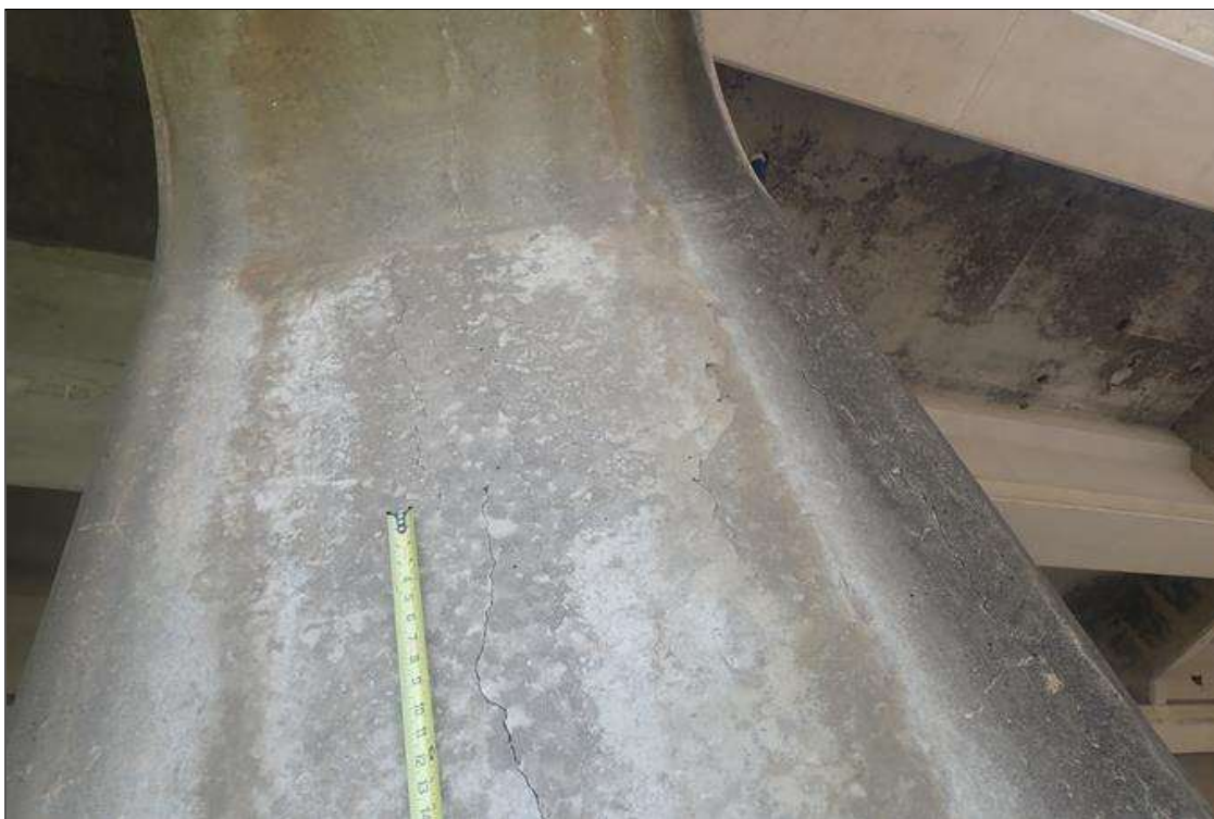
Bent 2 Pile 1: west face, multiple vertical cracks (up to 1/16 inch x full height) with delamination (2 feet wide) at top
