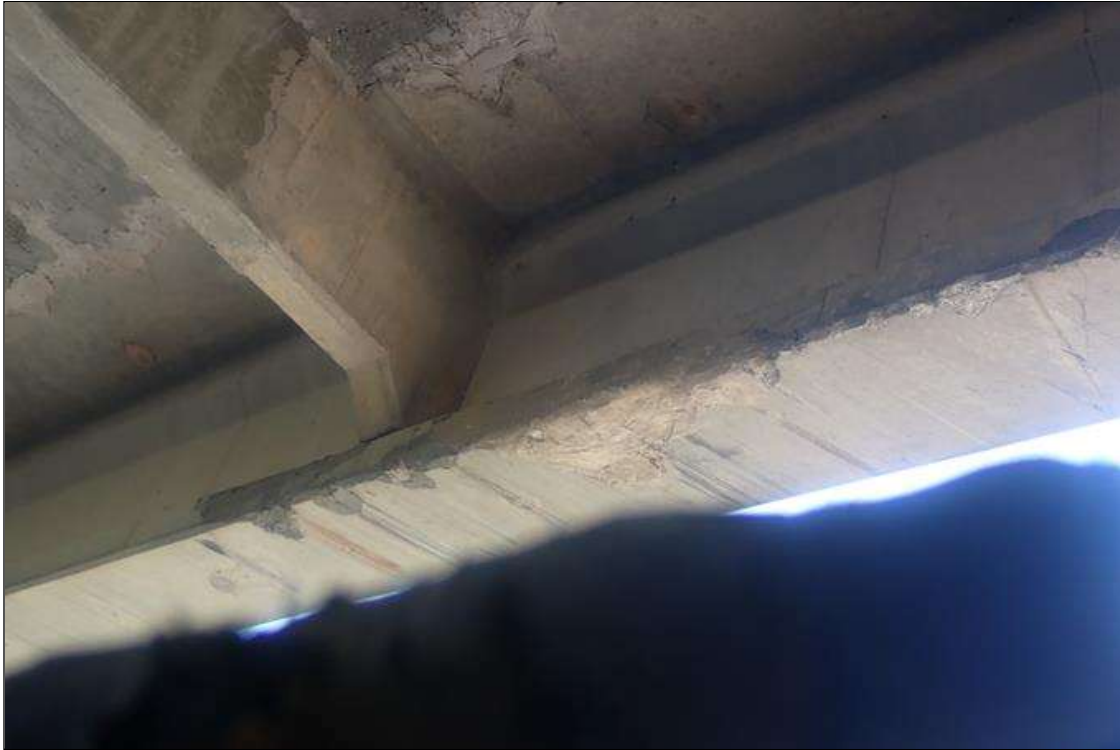
Span 3 Beam 1: 07-07-2023 no change since supplemental inspection, previously noted as: 2 FEET LONG X 10 INCHES HIGH PATCHED AREA OVERVIEW LOCATED 13 FEET FROM BENT 3 OVER SOUTHBOUND TRAVEL LANES
