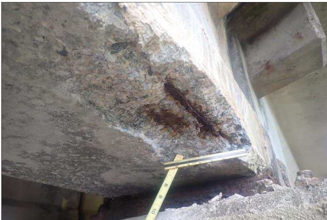
Span 3 Beam 4: (PAR) 1 foot from bent 3, bottom flange, right face, spall (16 inch x 7 high x 2 inch deep) with (1) broken strand and (1) rusted strand
