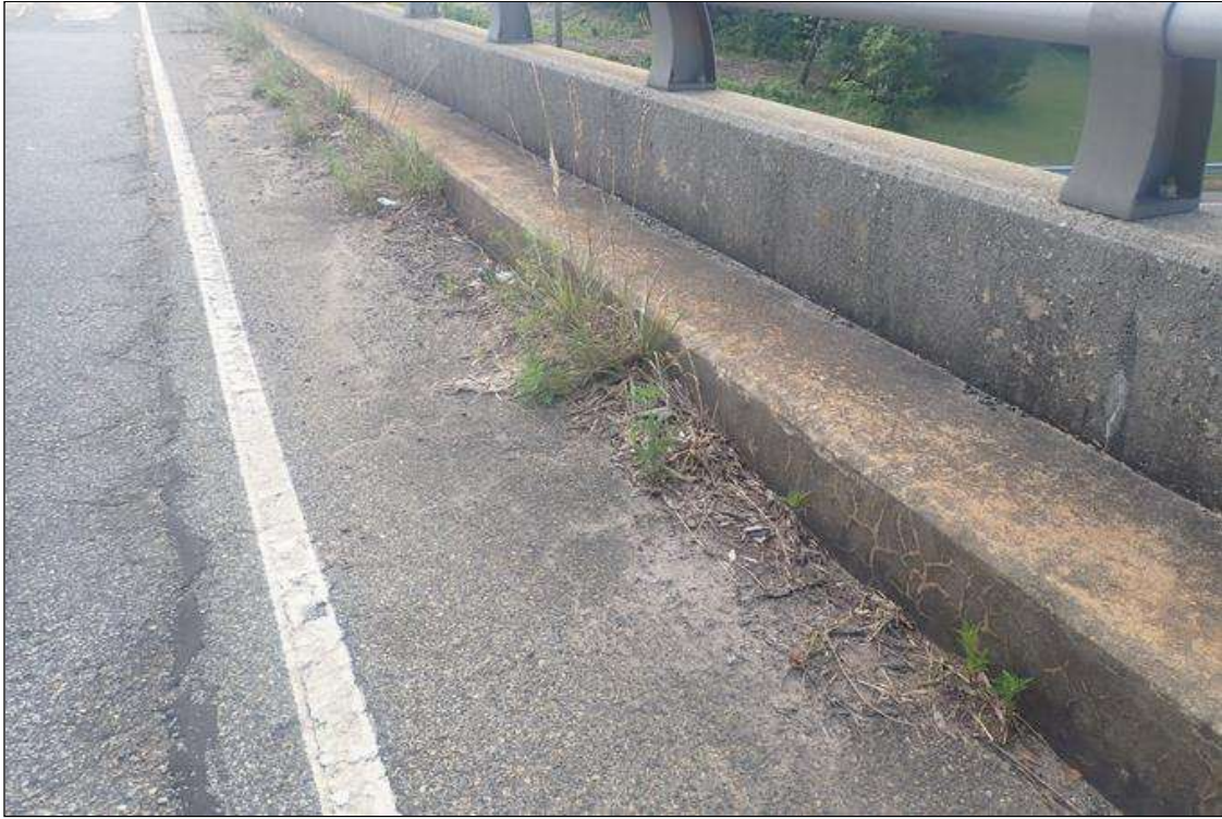
along both curbs, debris and vegetation, inhibits drainage
