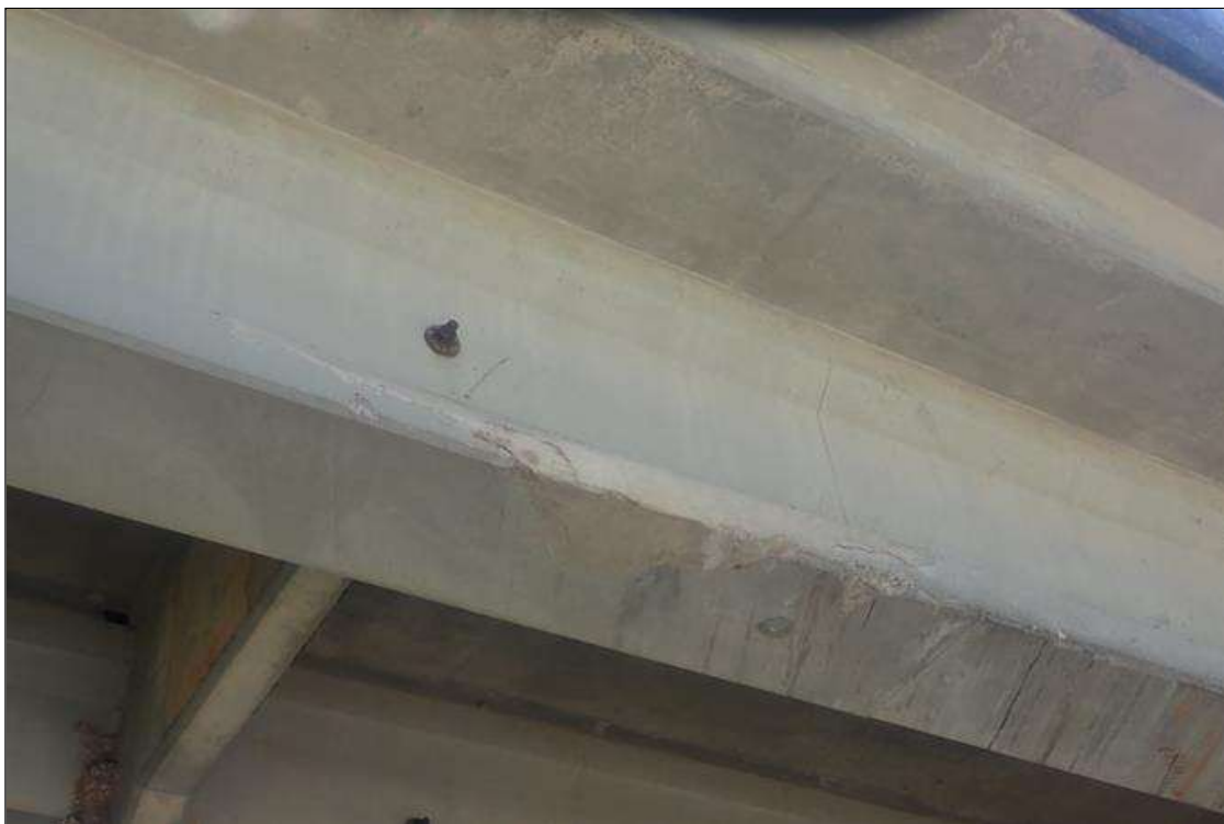
Span 3 Beam 4: 22 feet from bent 2, over left southbound lane, bottom flange right face, previous patch (approximately 8 feet long)
