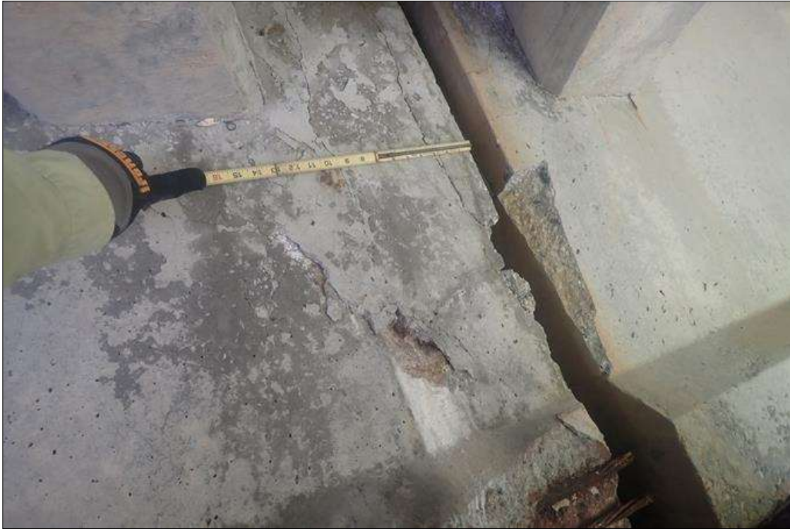
Span 3 Beam 3: (PAR) at bent 3, at right face, web, delamination/spall (16 inch x 30 inch x 1 inch deep) with cracks (up to 1/16 inch)
