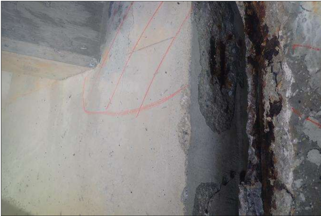
Span 4 Beam 3: at bent 3, end of web, spall/delamination (29 inch high x full width x up to 1.5 inch deep) with exposed rusted rebar extending along faces (up to 16 inches)
