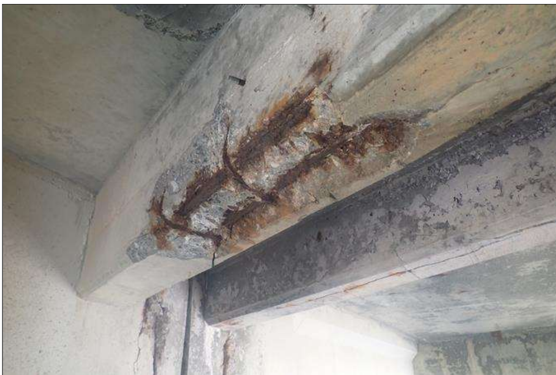
Span 3 Deck: bent 2 end diaphragm, bay 2, spall (4 feet x 8 inch x 2 inch) with exposed rusted rebar
