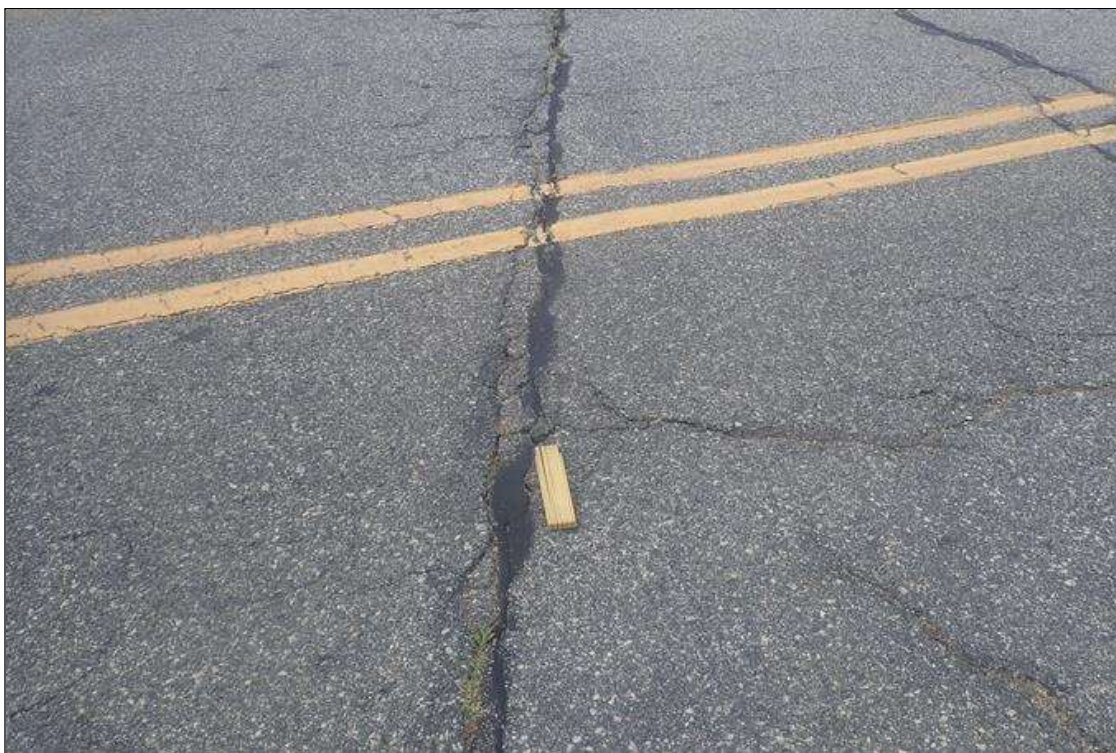
Span 4 Wearing Surface: 1/2 inch full length transverse crack at abutment 2
