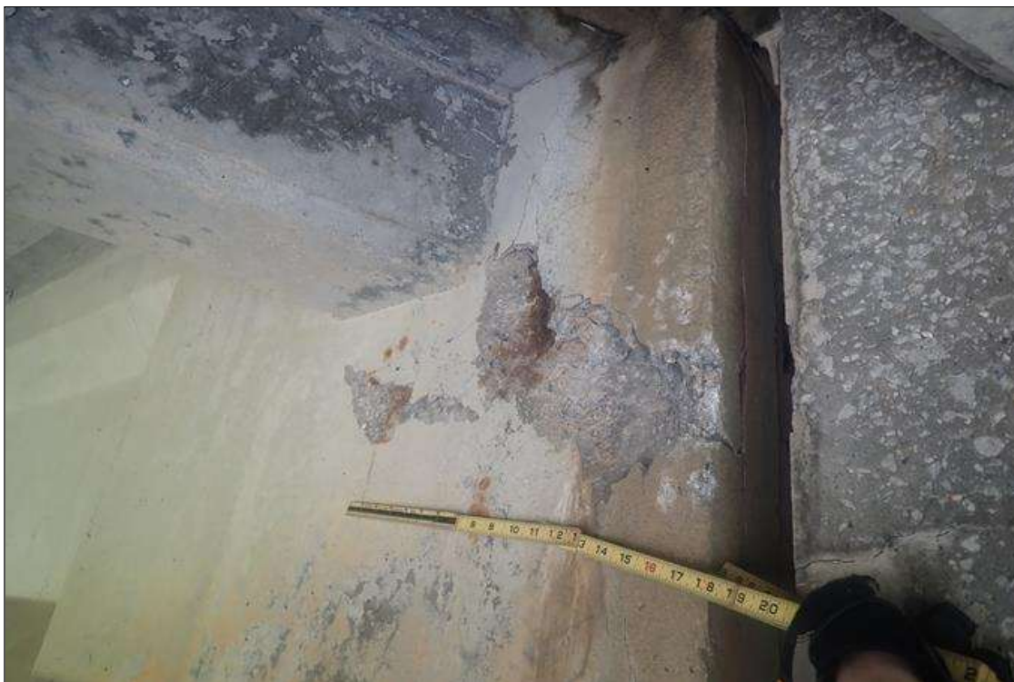
Span 1 Beam 3: (PAR) at bent 1, end of beam, both faces, spalls (up to 4 inch x 28 inch x 2.5 inch deep) with exposed rusted rebar
