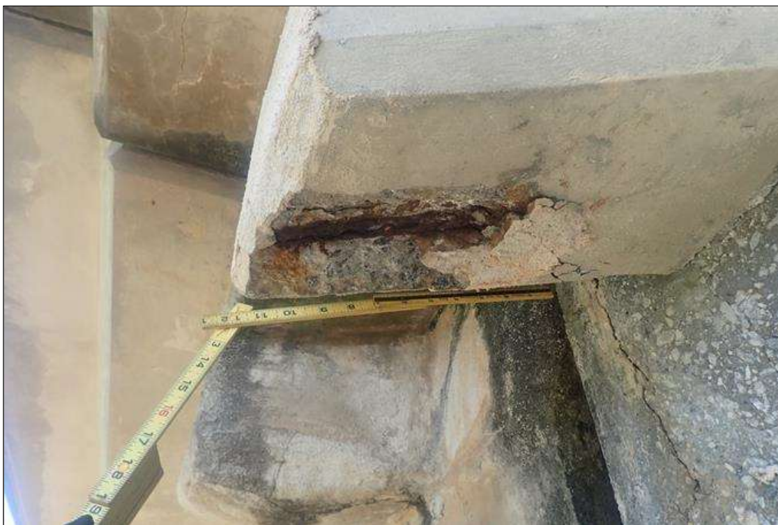
Span 3 Deck: bent 3 end diaphragm, left overhang, partially failed patch (12 inch x 6 inch x 1 inch deep) with exposed rusted rebar
