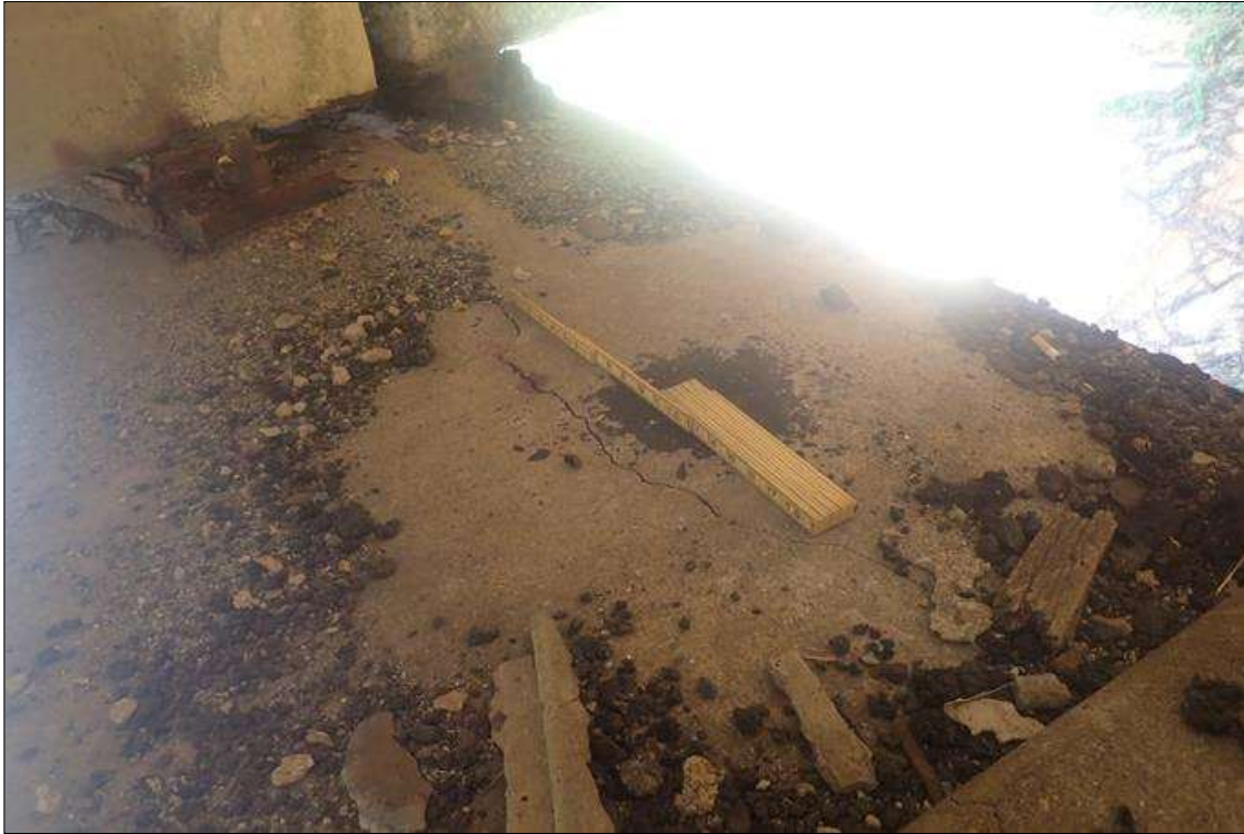
Bent 3 Cap 1: top face, bay 1, longitudinal crack (up to 1/8 inch x 7 feet)
