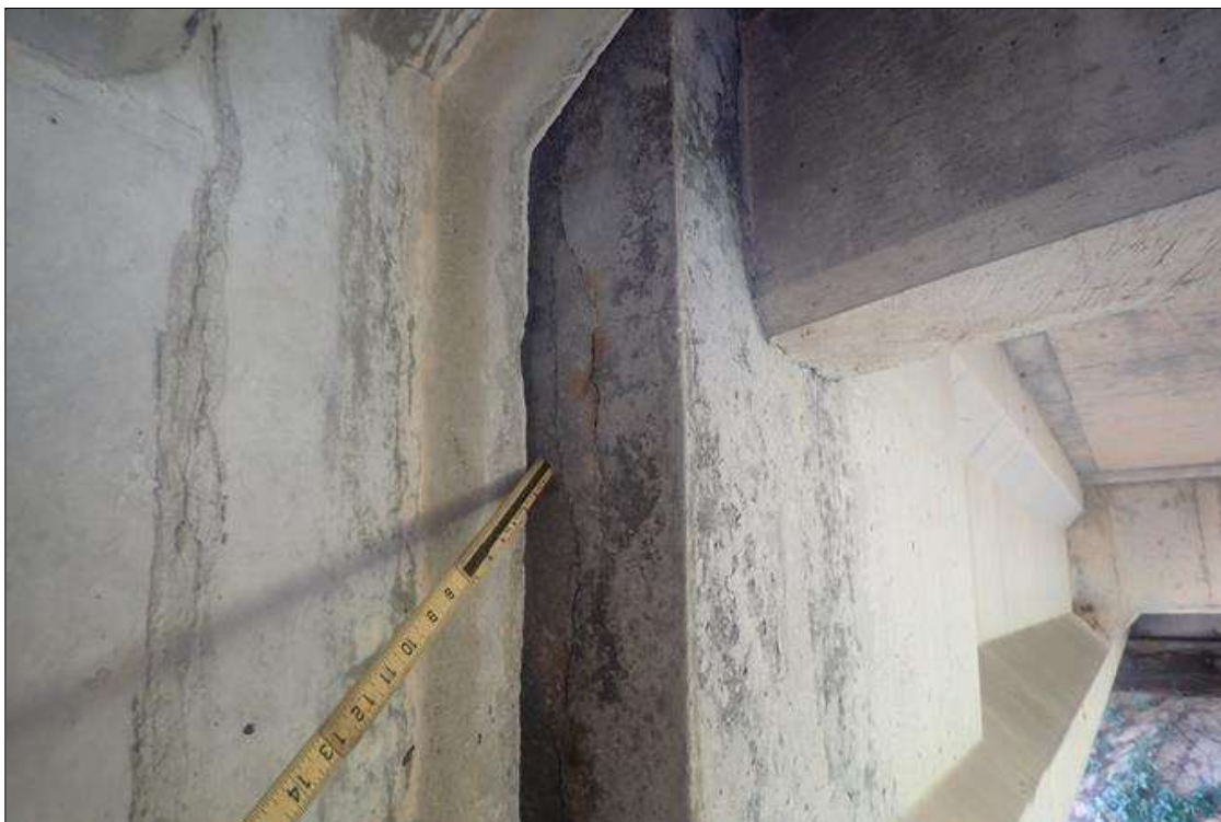
Span 4 Beam 2: (PAR) at bent 3, end of web, vertical crack (0.03 inch x 30 inch)
