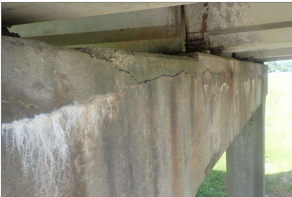
Bent 2 Cap 1: (PAR) HORIZONTAL CRACKING UP TO 1/4 INCH WITH DELAMINATIONS/SPALLS (UP TO 1 INCH DEEP), EFFLORESCENCE BUILDUP AND RUST STAINS AT TOP EDGE ALONG LENGTH OF BOTH FACES.
