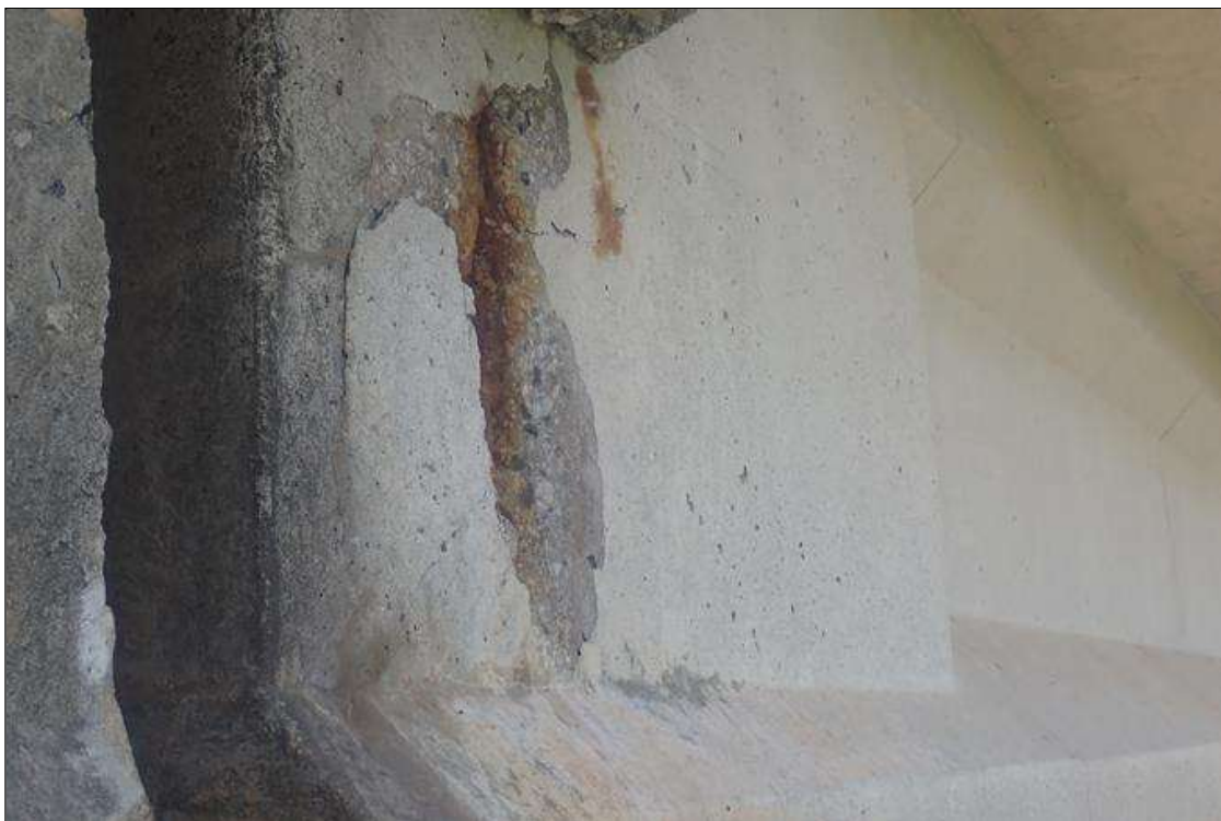
Span 1 Beam 1: 1 FOOT HIGH X 6 INCH LONG X 1 INCH DEEP SPALL ON LEFT SIDE WITH EXPOSED RUSTED REBAR OVER PIER 1.
