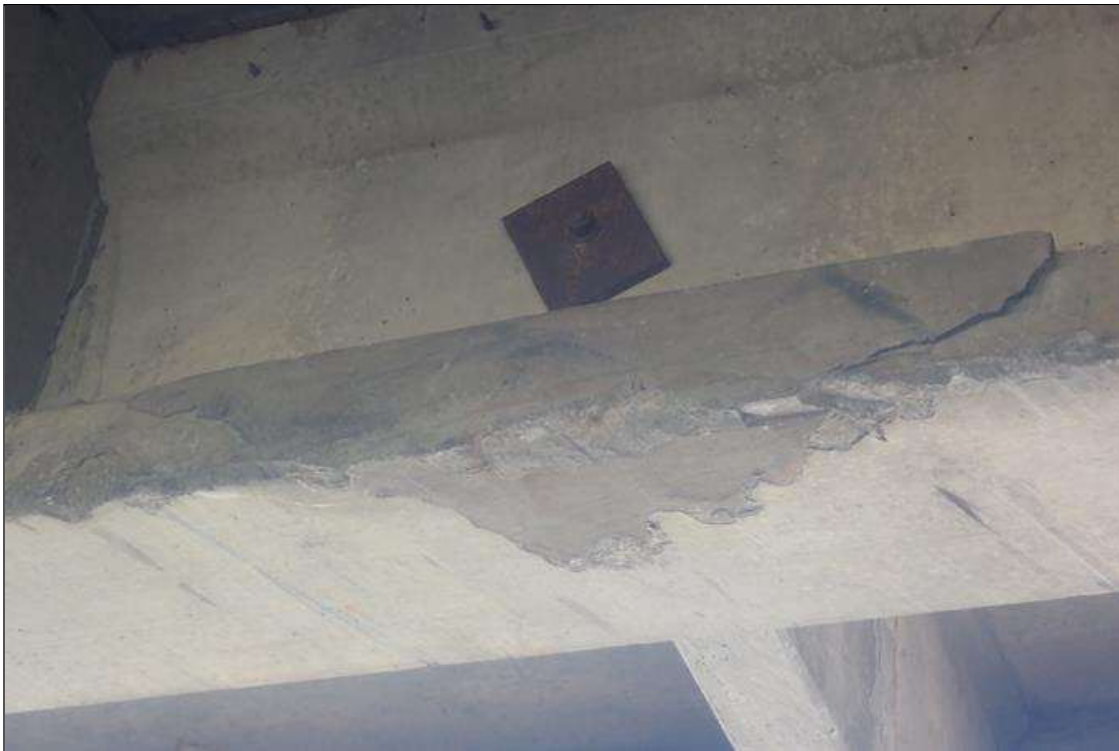
Span 3 Beam 2: (PAR) 07/07/2023 no apparent change since supplemental inspection, located at previous repair (5 feet long), previously noted as: IMPACT DAMAGE - LOCATED 14 FEET 1 INCH FROM BENT 3 ; DIMENSIONS ARE 2 FEET 6 INCHES LONG X 4 INCHES HIGH X 1/2 INCH DEEP
