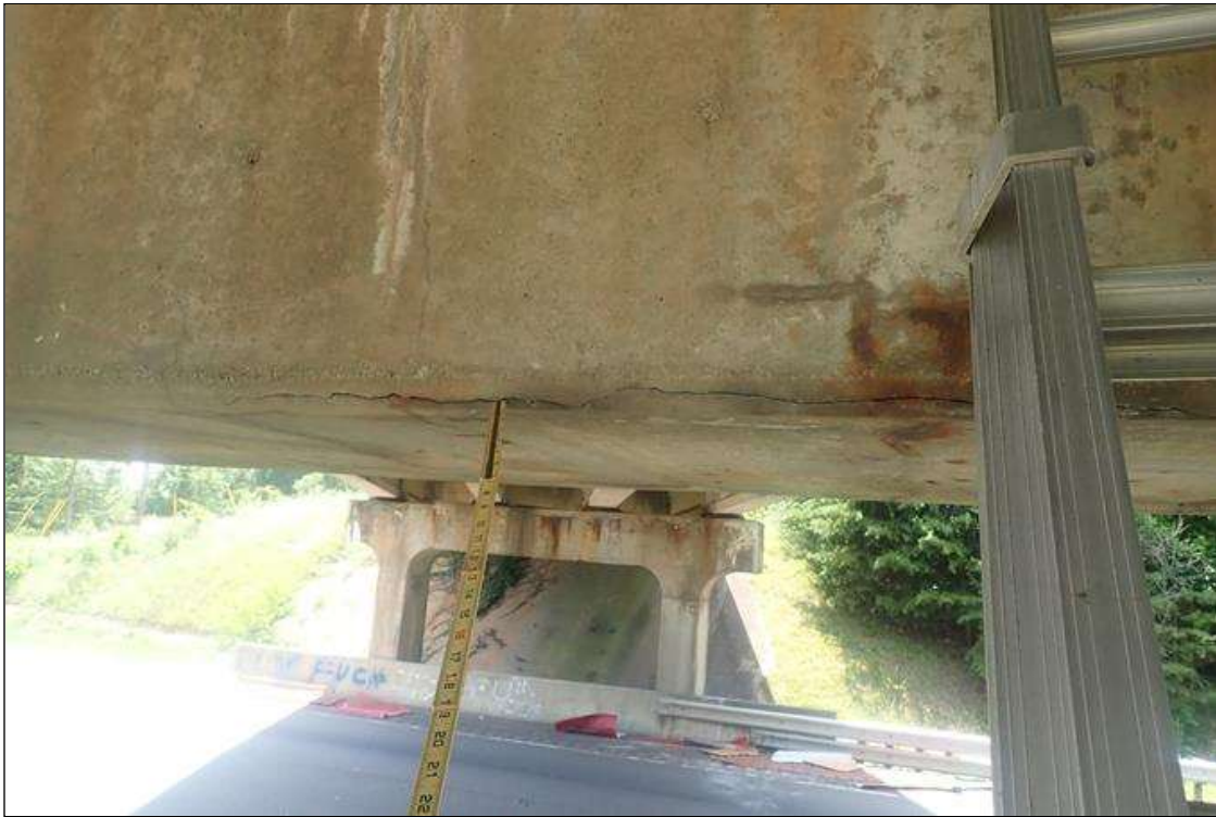
Bent 2 Cap 1: (PAR) south face, below bay 2, bottom corner, longitudinal crack (1/16 inch x 9.5 feet) with rust stains, and spall/delamination (3 feet x 1 foot x 2 inch deep) with exposed rusted rebar
