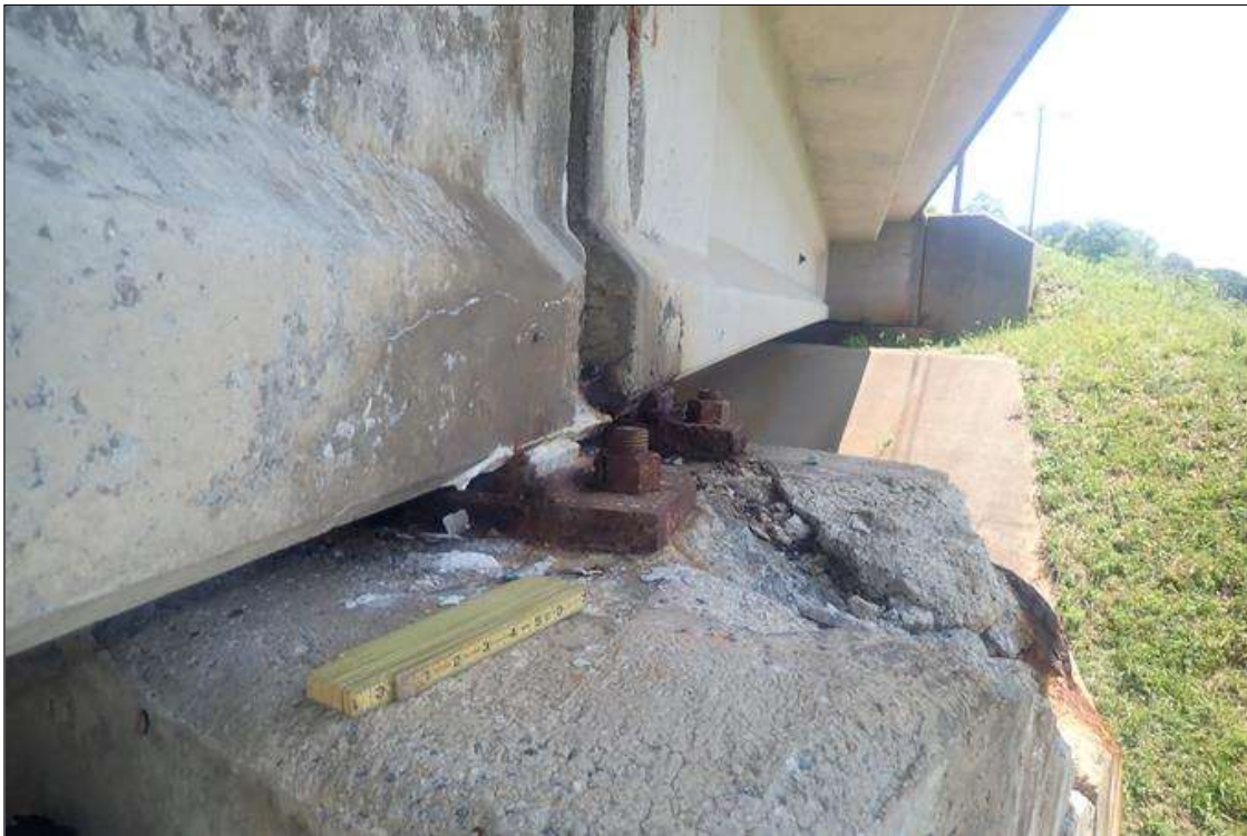
Bent 1 Cap 1: (PAR) west end of cap, delaminated/partially failed previous repair (3.5 feet long x full height x full width), with spalls (up to 2 feet x 16 inch x 2 inch deep) with exposed rusted rebar, rust stains, efflorescence buildup, and cracks (up to 1/8 inch)
