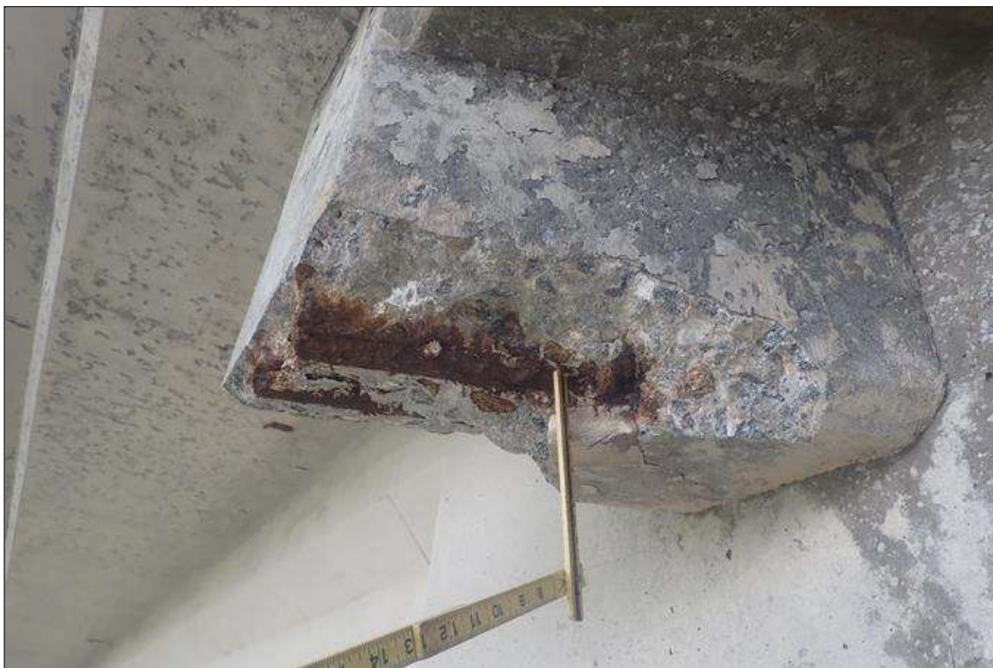
Span 1 Deck: bent 1 end diaphragm, right overhang, spall (12 inch x 8 inch x 2 inch deep) with exposed rusted rebar
