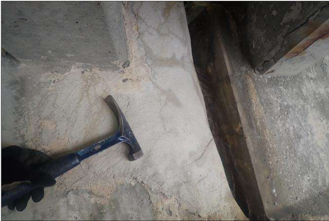
Span 3 Beam 4: FULL HEIGHT X 2 FEET LONG PATCHED AREA THAT IS SOUND WITH CRACKS UP TO 1/32 INCH ON LEFT SIDE WEB OVER PIER 2.
