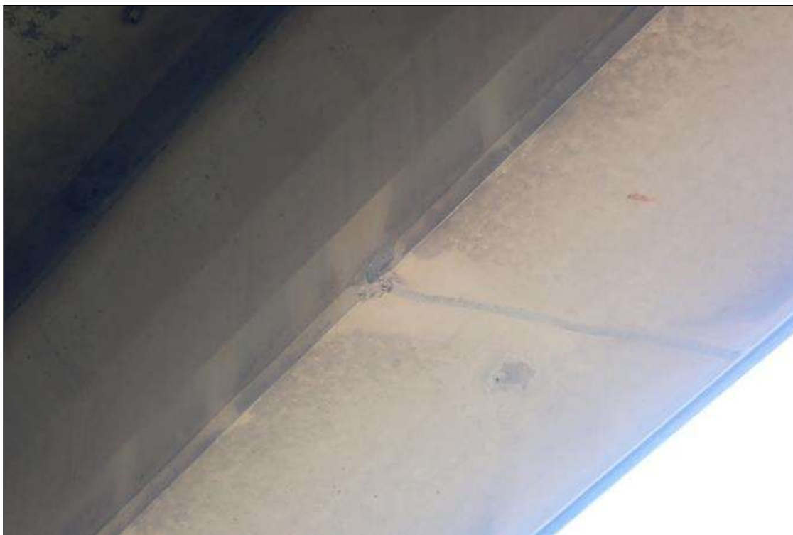
Span 2 Beam 1: CHIPPED AREA ALONG BOTTOM EDGES OF FLANGE UP TO 3 INCH X 3 INCH X 1/2 INCH DEEP FROM IMPACT DAMAGE AT MIDSPAN.
