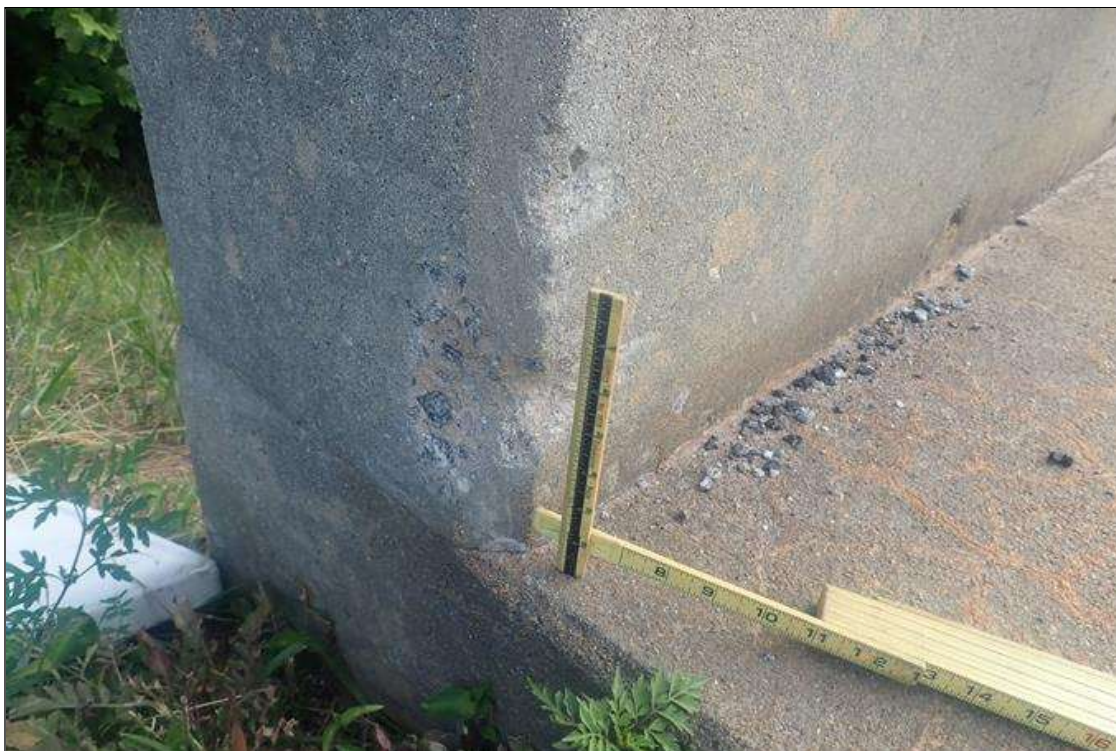
Span 4 Right Bridge Rail: concrete end post, spall (4 inch x 2 inch x 1/2 inch deep)
