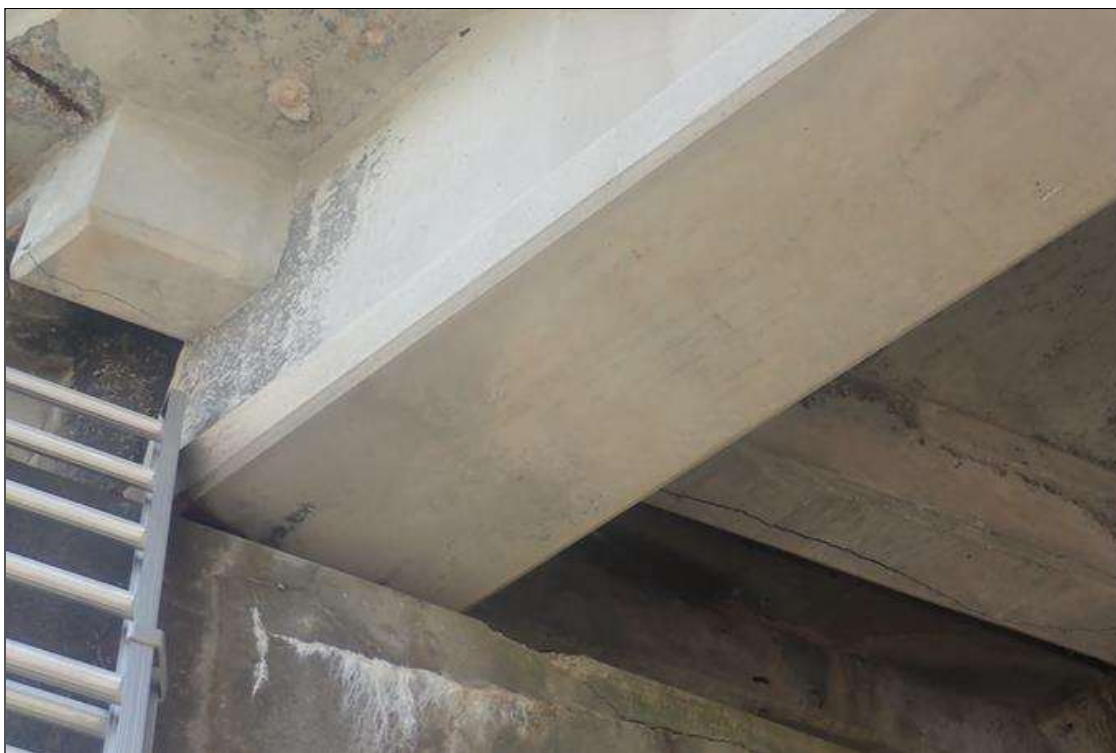
Span 2 Deck: (PAR) bent 2 end diaphragm, longitudinal crack (up to 1/4 inch x full length) with rust stains
