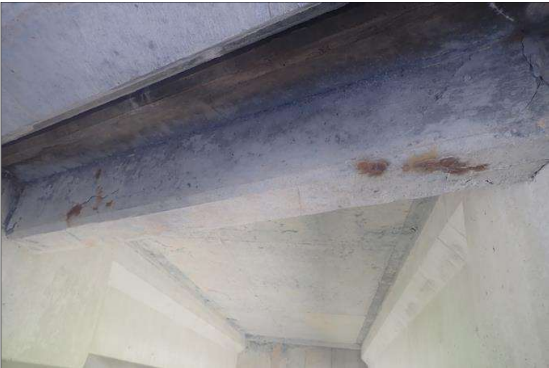
Span 1 Deck: (PAR) bent 1 end diaphragm, bay 2, longitudinal crack (up to 1/16 inch x 7 feet) with rust stains
