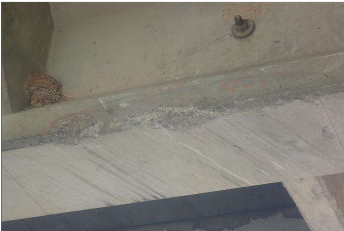
Span 3 Beam 3: (PAR) IMPACT DAMAGE - LOCATED 16 FEET 4 INCHES FROM BENT 3 - DIMENSIONS ARE 2.833 FEET LONG X 5 INCHES HIGH X 1 INCH DEEP ALONG NORTH EDGE OF BOTTOM FLANGE - 07/07/2023 no apparent change from supplemental inspection
