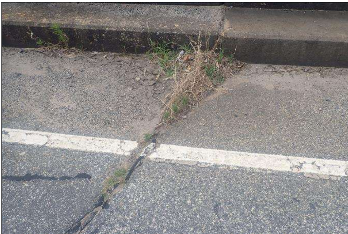
Span 4 Expansion Joint: DEBRIS IMPACTION AND VEGETATION GROWTH IN JOINT AT BOTH GUTTERLINES FOR FIRST 3 FEET
