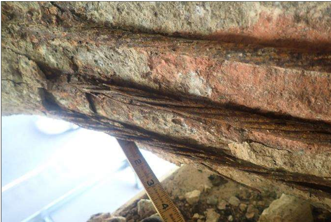
Span 2 Beam 2: (PAR) at bent 2, right face, bottom flange, spall (3.5 feet x 11 inch x 2 inch deep) with (2) broken strands and (1) rusted strand; similar left face
