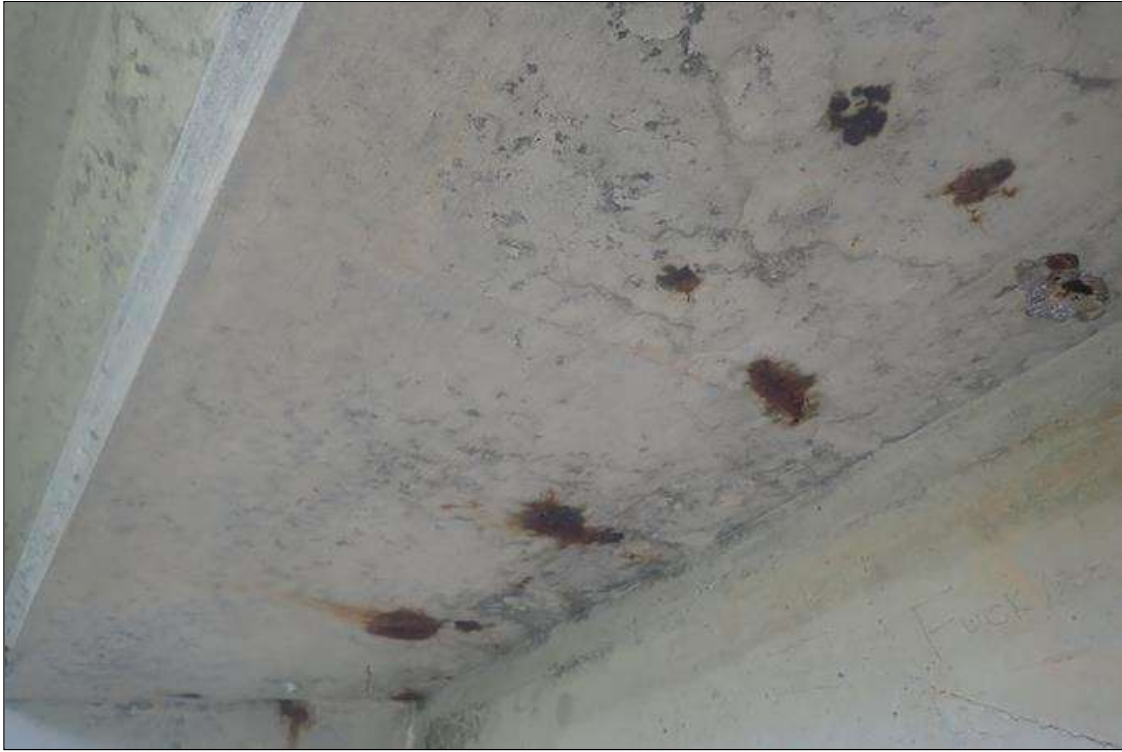
Span 1 Deck: (PAR) underside, at random, areas of transverse/map cracks (hairline) with rust stains
