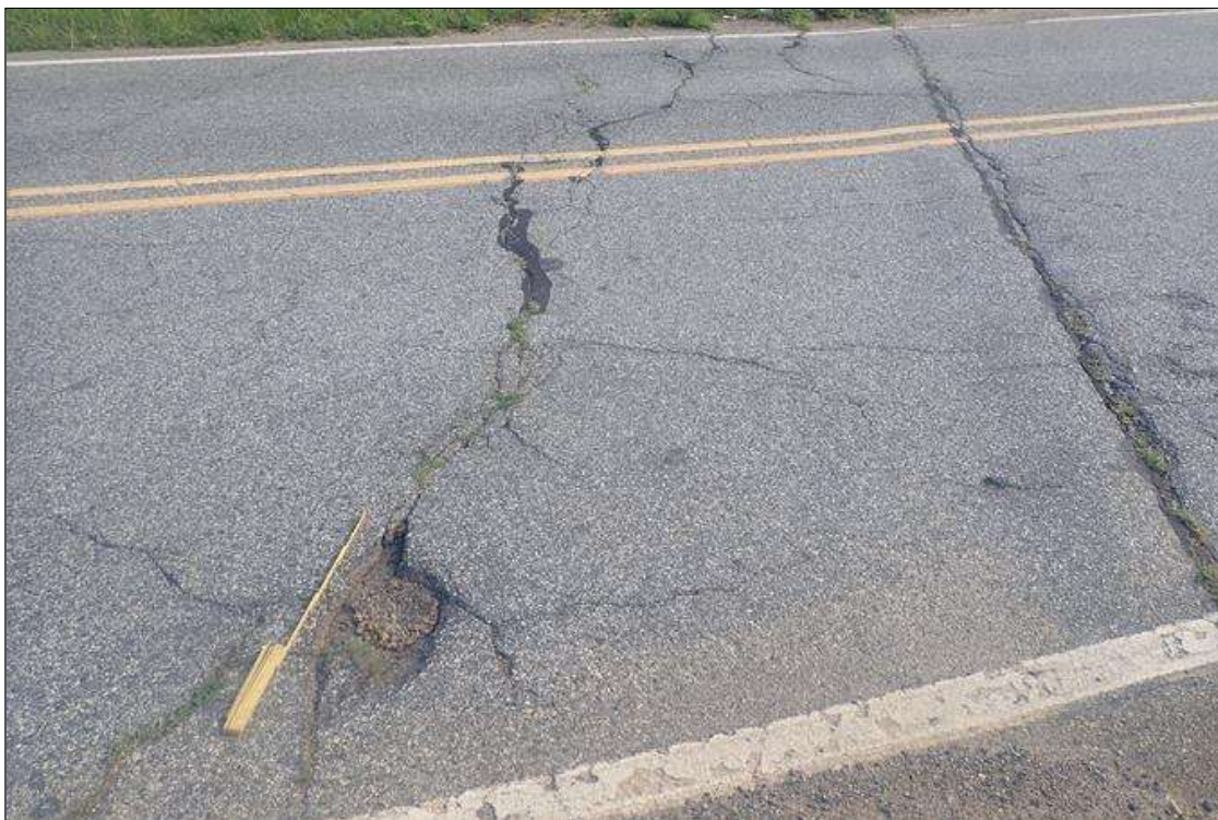
north approach asphalt, at bridge, transverse/map cracks (up to 1/2 inch); southbound lane, pothole (2 feet x 1 foot x 2 inch deep)
