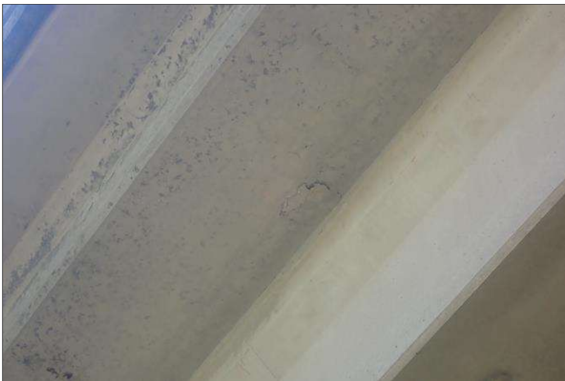
Span 1 Deck: underside, right overhang, midspan, delamination (6 inch diameter)
