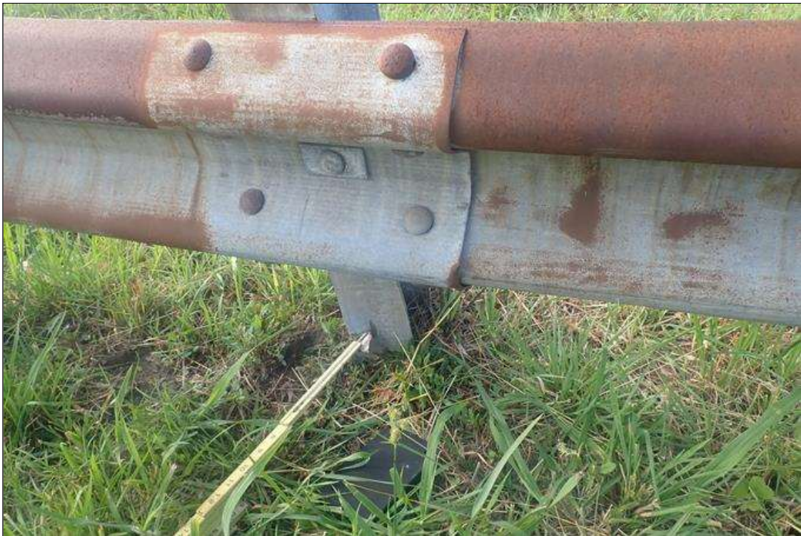
(PAR) northwest guardrail, at center, improper lap and torn post
