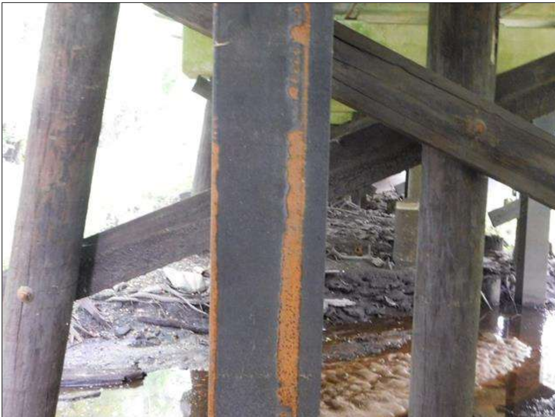
Bent 2 Pile 2 (Crutch Bent): SCATTERED AREAS OF SURFACE RUST (14 FT.)
