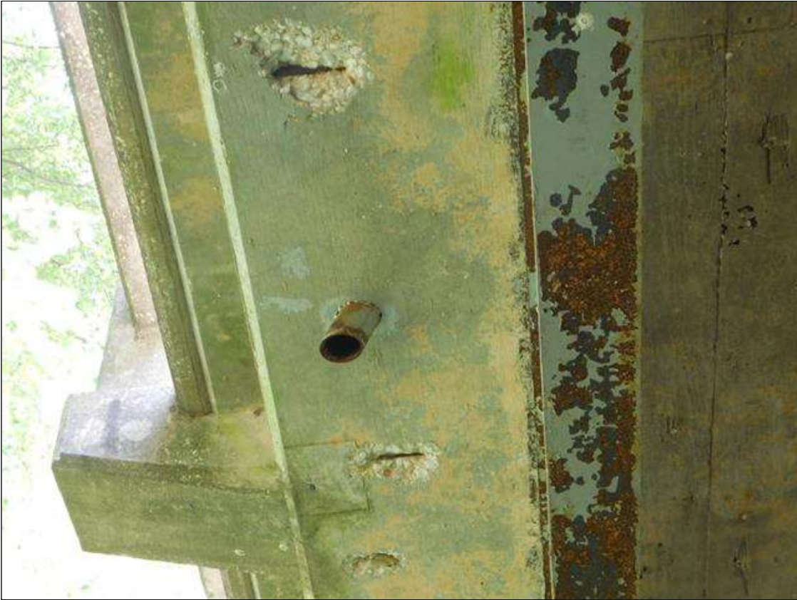
Span 3 Deck: (3) SPALLED AREAS WITH REBAR VISIBLE IN SCATTERED LOCATIONS. BOTTOM OF LEFT OVERHANG. AREAS AREA UP TO: 10" DIAMETER x 2" DEEP
