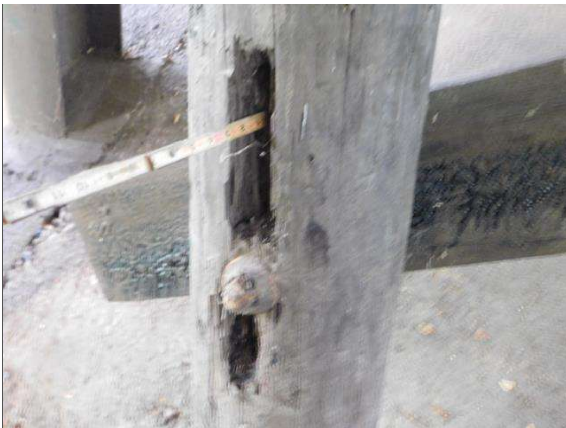
Bent 1 Pile 4: 17" TALL x 3" WIDE x 2" DEEP AREA OF 100% SECTION LOSS ON NORTH FACE AT LOWER CROSS-BRACE
