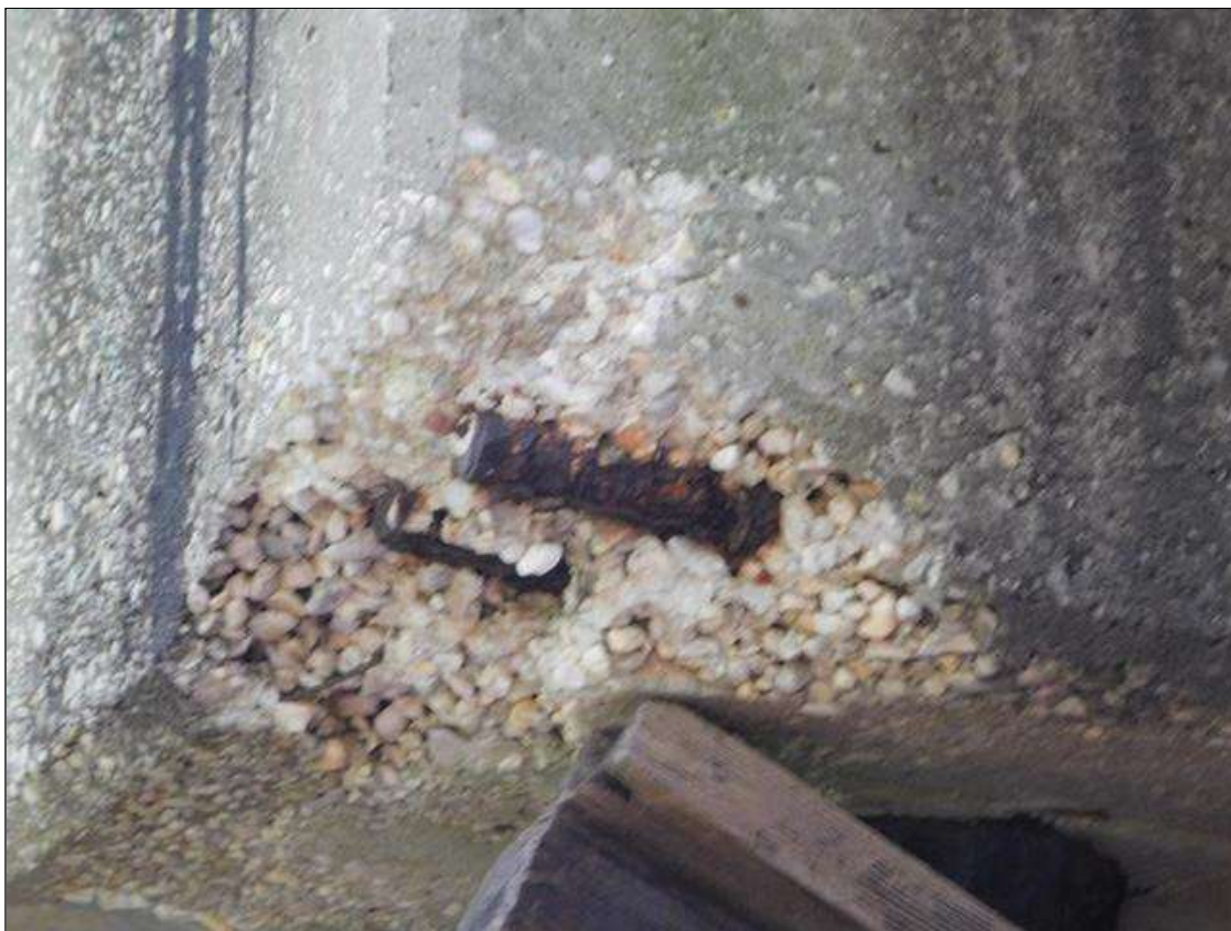
Bent 2 Cap 1: BOTTOM SOUTHWEST CORNER HAS A 14" x 10" x UP TO 7" DEEP SPALL WITH (2) MAIN REBAR EXPOSED. "PAR" ISSUED
