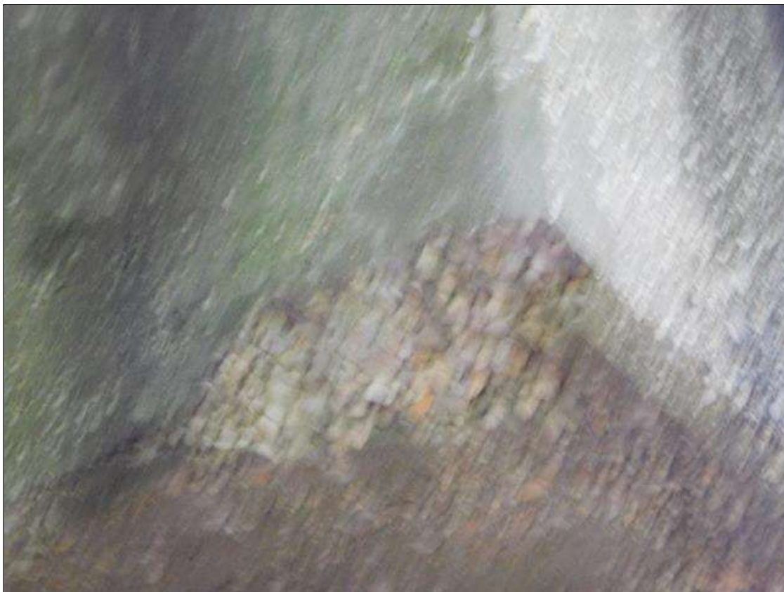
Bent 2 Cap 1: 12" x 6" x 2" DEEP SPALL IN BOTTOM NORTHWEST CORNER
