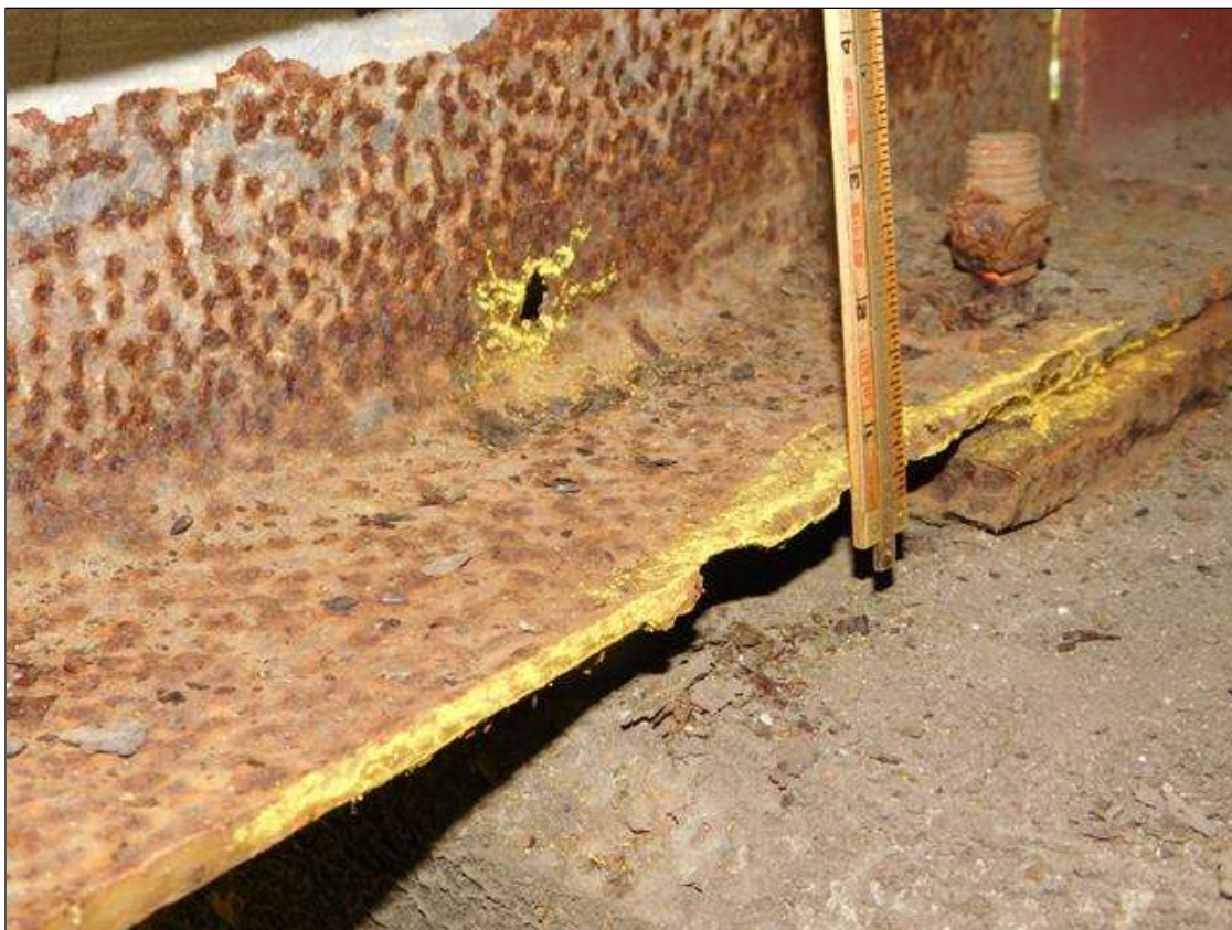
Span 1 Beam 1: RIGHT BOTTOM FLANGE OVER BENT 2 HAS A AREA OF SECTION LOSS WITH DOWN TO KNIFE'S EDGE REMAINING. AREA IS: 11" LONG x 3" WIDE. "PAR" ISSUED
