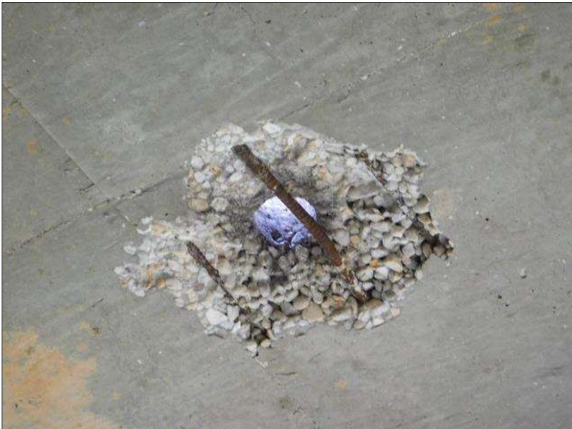
Span 2 Deck: 2' DIAMETER x UP TO 3" DEEP SPALL WITH (3) REBAR EXPOSED. BOTTOM OF DECK BAY 4 AT MID-SPAN. "PAR"
