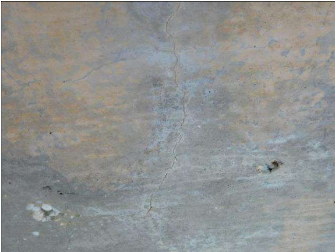
Span 1 Deck: INTERMITTENT FULL WIDTH X 1/32" WIDE TRANSVERSE CRACKS WITH EFFLORESCENCE IN THE UNDERSIDE OF THE DECK AT 1' TO 3' SPACING
