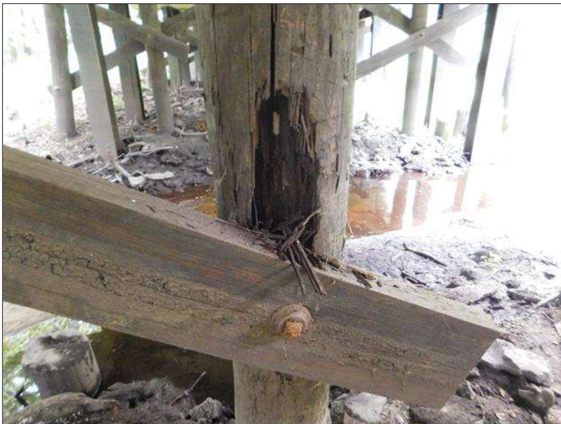
Bent 2 Pile 4: 24" TALL x 8" WIDE x 3" DEEP AREA OF DECAY IN SOUTH FACE AT LOWER CROSS-BRACE. "PAR ISSUED
