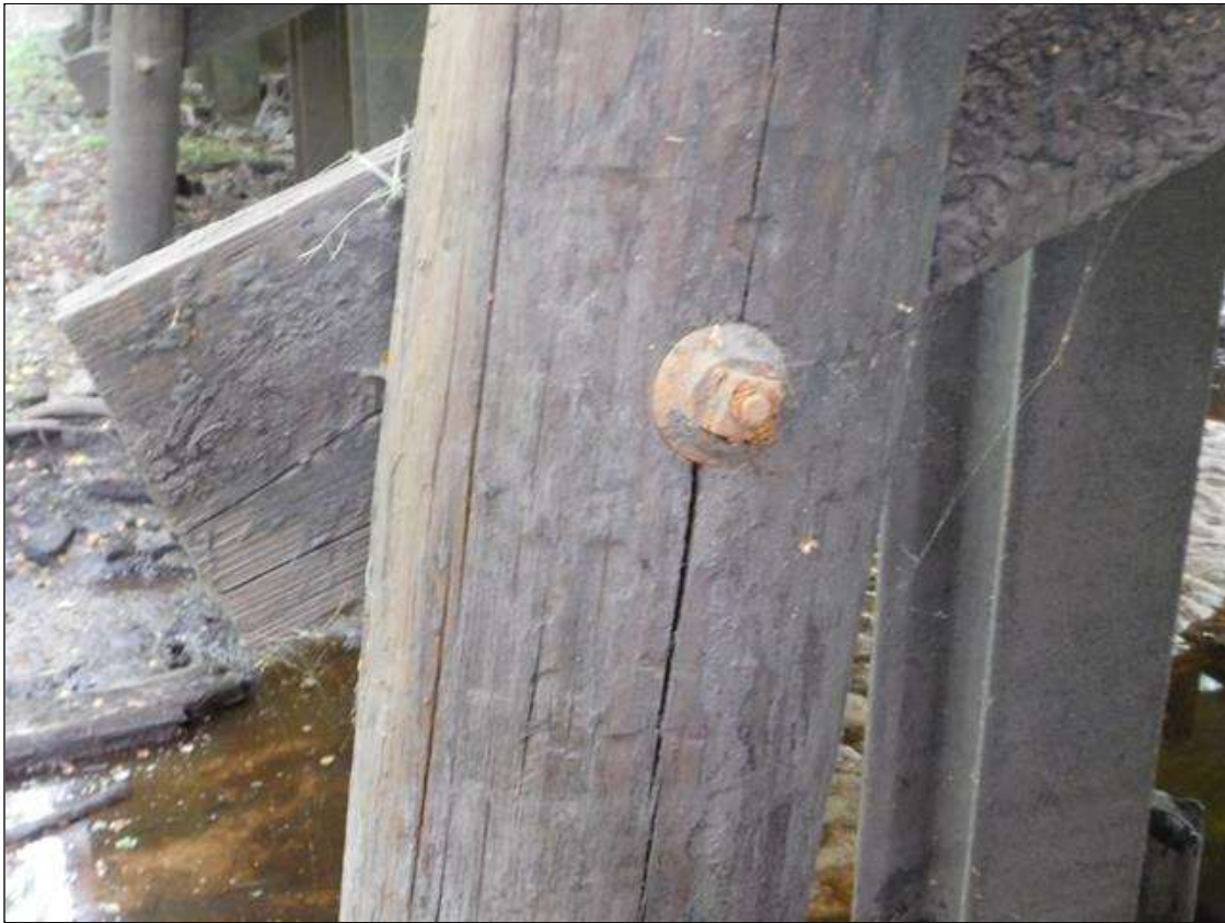
Bent 2 Pile 1: SCATTERED CHECKS UP TO 1/4" WIDE
