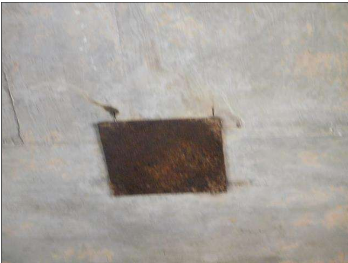
Span 3 Deck: METAL PLATE BOLTED TO BOTTOM OF DECK IN BAYS 1 AND 3 AT BENTS 2 AND 3.
