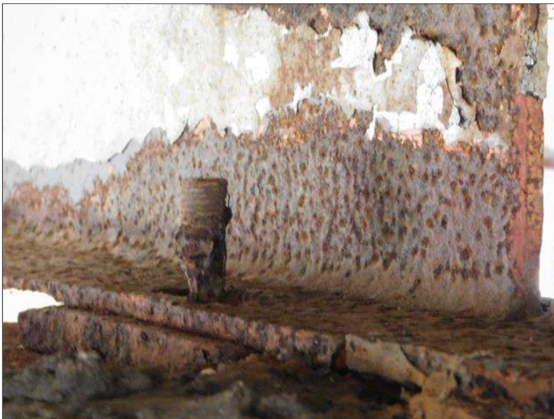
Span 5 Beam 3 - Near Bearing: ANCHOR BOLT NUT MISSING ON BOTH SIDES. "PAR"
