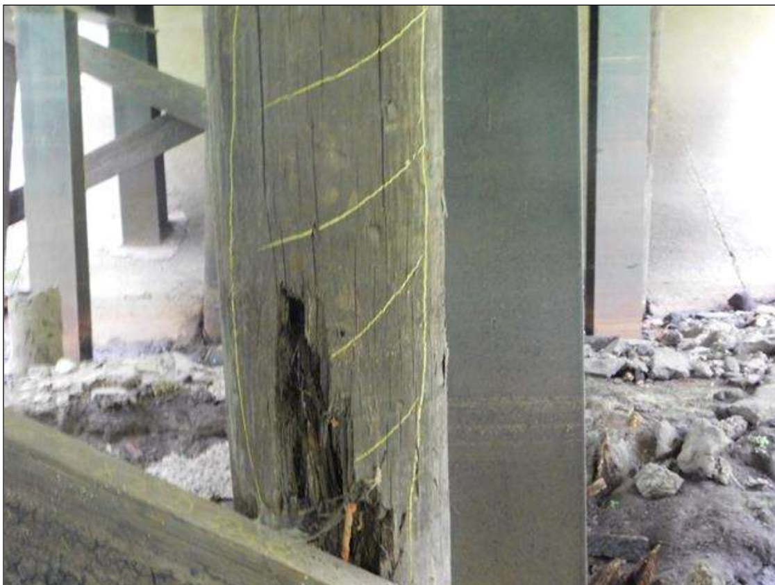
Bent 4 Pile 4: SOUTH FACE HAS A AREA OF DECAY WITH ADJACENT HOLLOW SOUNDS. AREA IS: FROM BOTTOM OF CAP DOWN 6' x 10" x 3" DEEP. "PAR"
