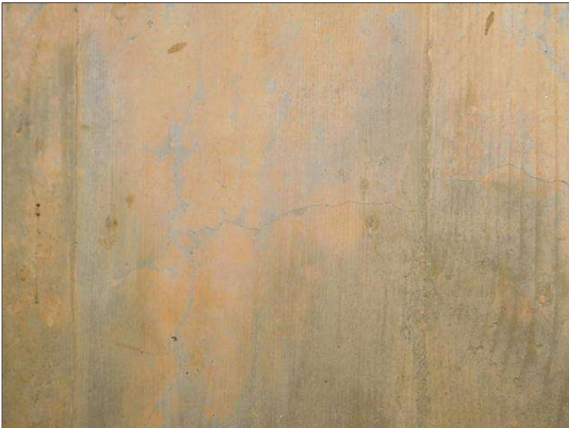
End Bent 2 Abutment: SCATTERED AREAS OF HAIRLINE MAP CRACKING
