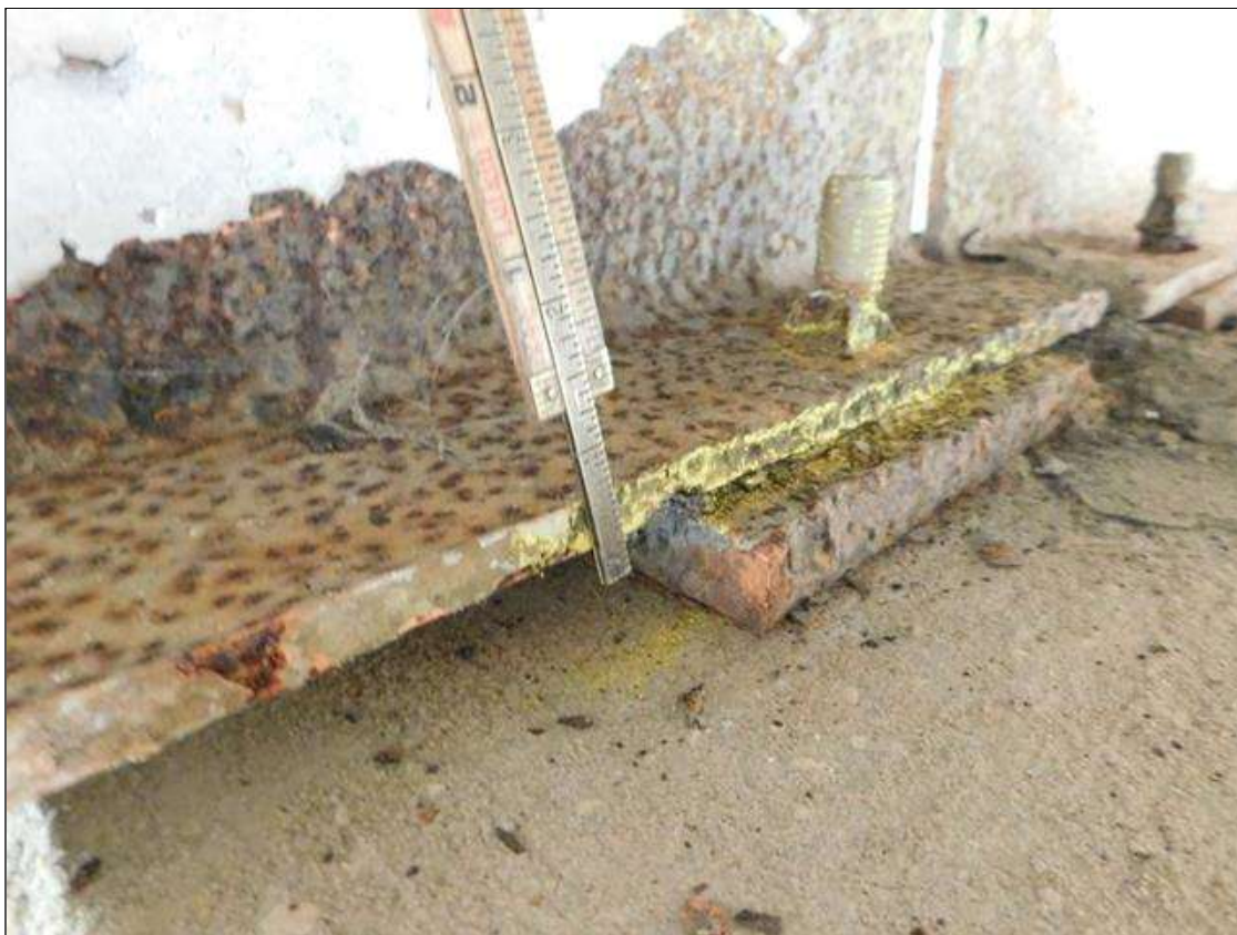
Span 3 Beam 3: RIGHT BOTTOM FLANGE OVER BENT 4. HAS A AREA OF SECTION LOSS WITH 1/4" REMAINING. AREA IS: 12" LONG x FULL WIDTH. "PAR"
