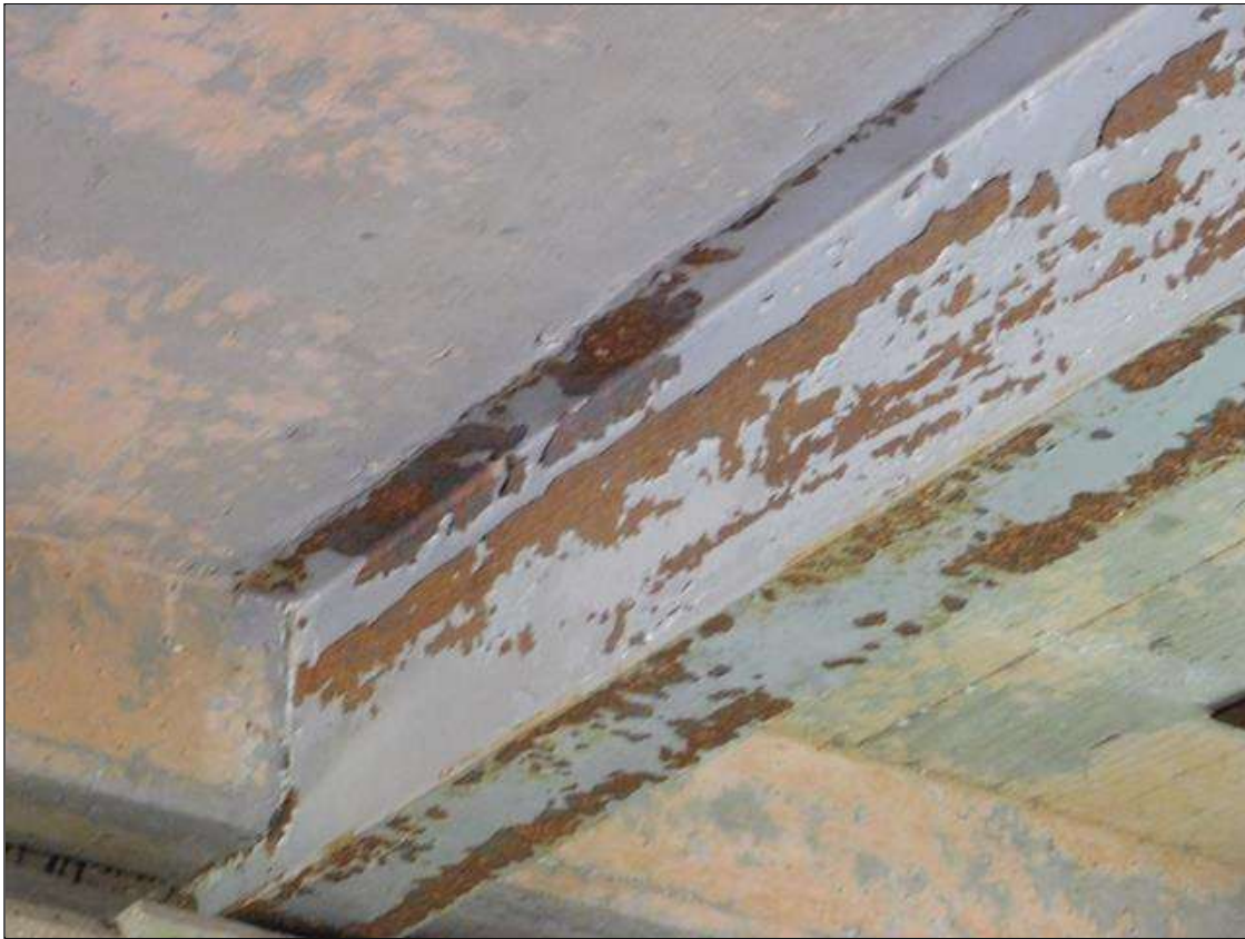
Span 5 Beam 2: SCATTERED AREAS OF RUST AND FLAKING IN BOTH FLANGES AND WEB
