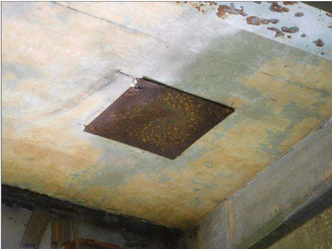
Span 3 Deck: 1'-4" LONG X 1'-4" WIDE PATCHED AREA WITH A STEEL PLATE IN BAY 4 AT BENT 2 / SIMILAR AT BENT 3
