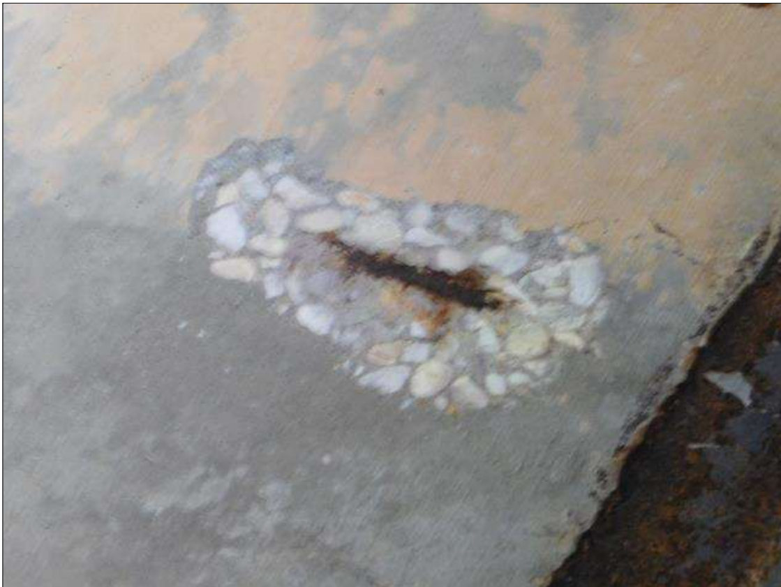
Span 5 Deck: 8" x 6" x 1 1/2" DEEP SPALL WITH REBAR EXPOSED IN BOTTOM OF DECK IN BAY 3, 4' FROM BENT 5
