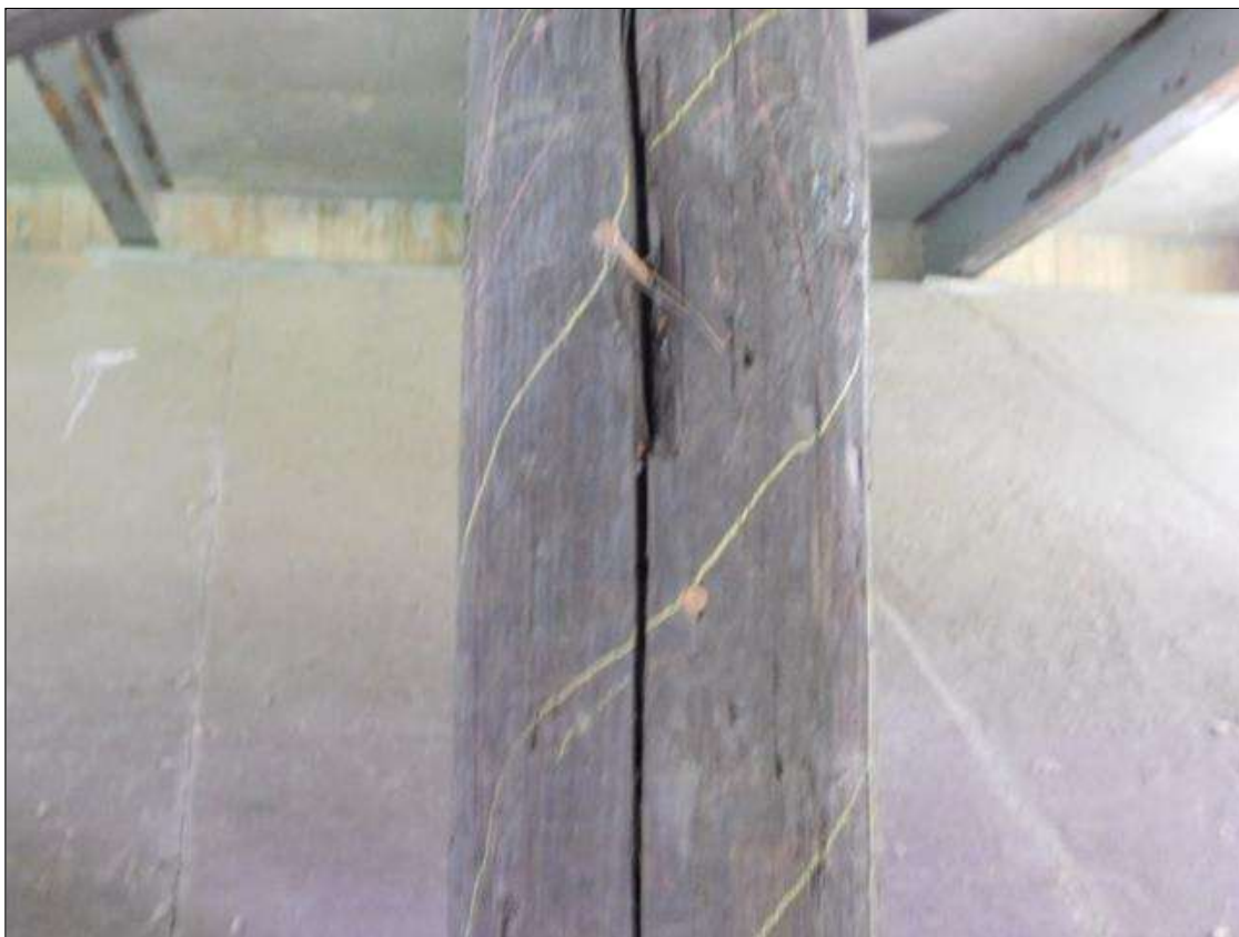
Bent 5 Pile 4: SOUTH FACE FROM BOTTOM OF CAP DOWN 5' x 1/2 CIRCUMFERENCE IS HOLLOW SOUNDING WITH A 10" x 1 1/2" x 2" DEEP AREA OF DECAY
