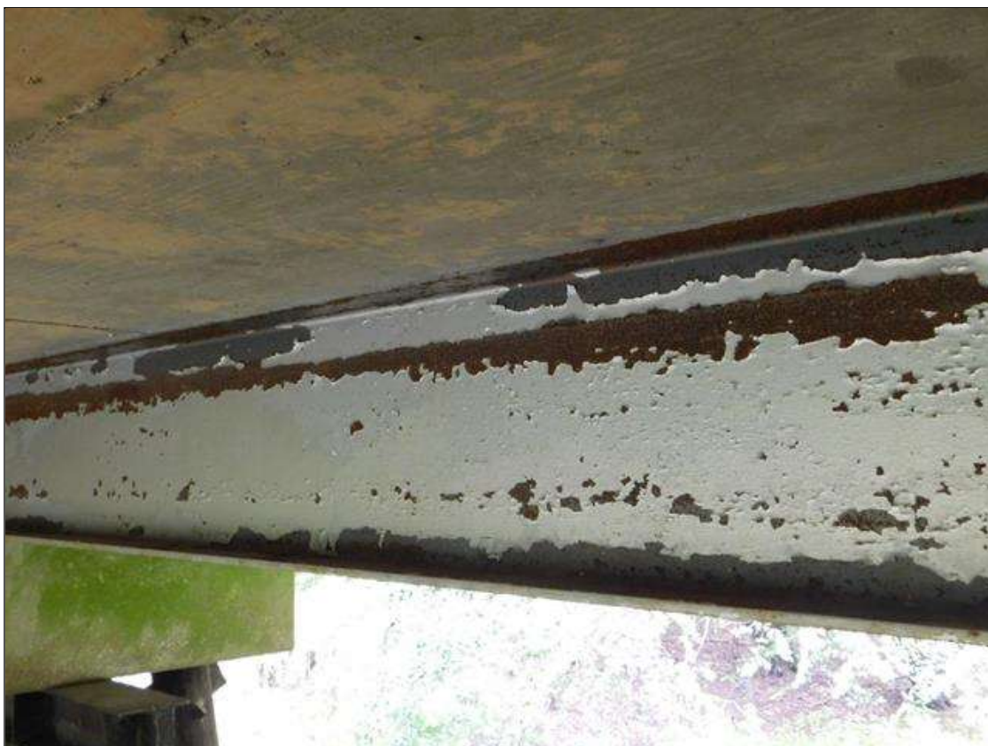
Span 3 Beam 2: SCATTERED AREAS OF RUST AND FLAKING IN BOTH FLANGES AND WEB
