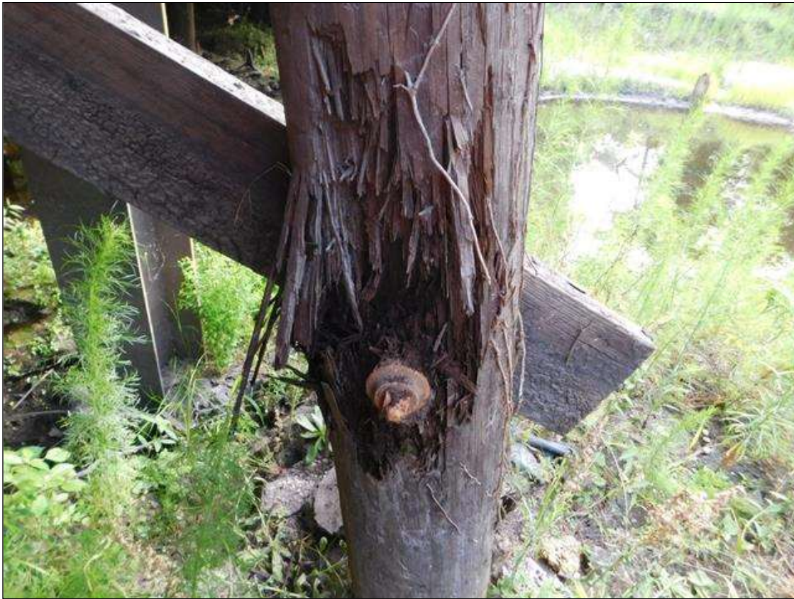
Bent 2 Pile 9: 2' TALL x 1/2 CIRCUMFERENCE x 3" DEEP AREA OF HEAVY DECAY ON SOUTH FACE AT LOWER CROSS-BRACE. "PAR"
