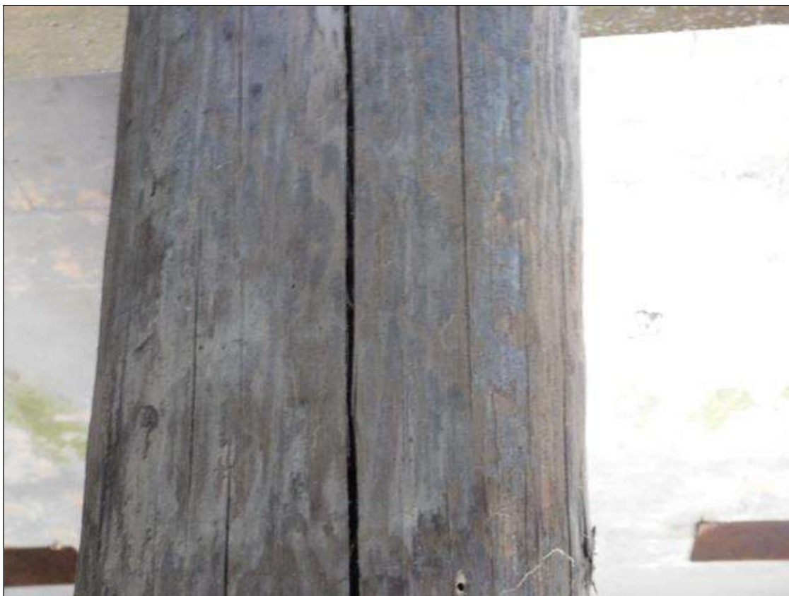
Bent 4 Pile 7: SCATTERED CHECKS UP TO 1/4" WIDE
