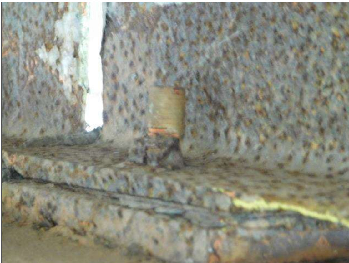
Span 3 Beam 4 - Far Bearing: LEFT ANCHOR BOLT NUT MISSING. "PAR"
