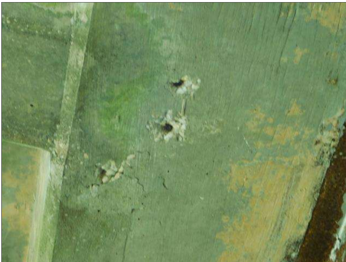
Span 4 Deck: (3) SPALLS UP TO 3" DIAMETER x 1" DEEP WITH REBAR VISIBLE AND ADJACENT 8" DIAMETER AREA OF DELAMINATION IN BOTTOM OF LEFT OVERHANG 4' FROM BENT 3.
