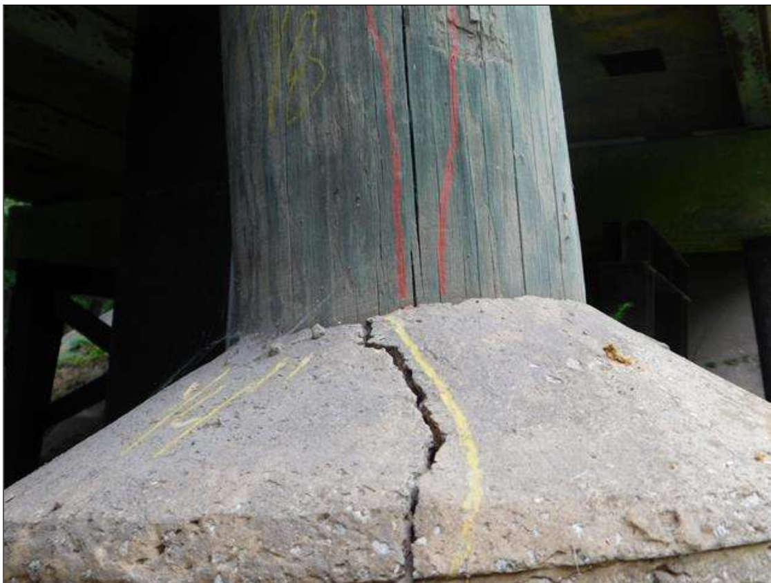
Bent 4 Pile 9: SCATTERED CHECKS UP TO 1/8" WIDE AND A CONCRETE ENCASEMENT THAT HAS SCATTERED CRACKS UP TO 1/4" WIDE
