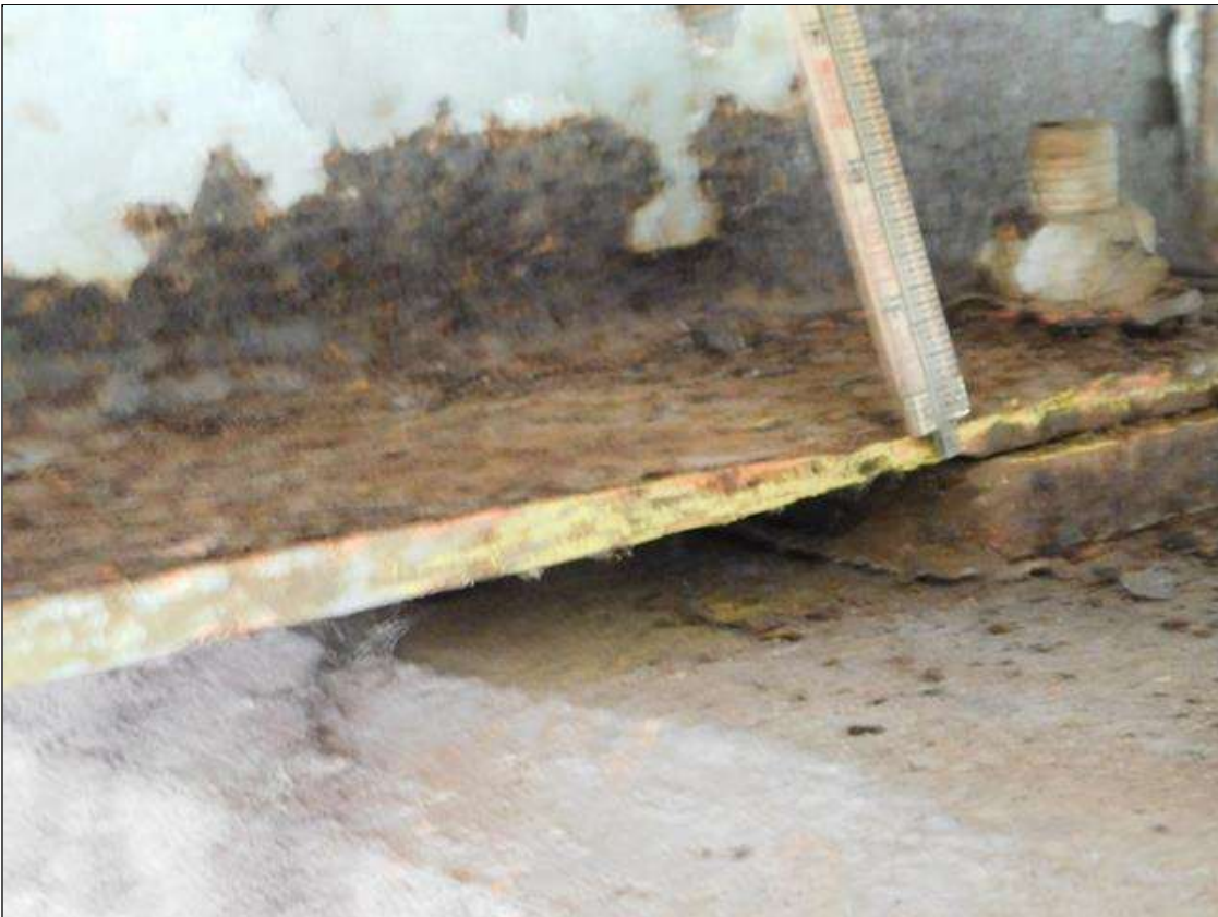
Span 1 Beam 4: RIGHT BOTTOM FLANGE OVER BENT 2. HAS A AREA OF SECTION LOSS WITH 1/4" REMAINING. AREA IS: 10" LONG x 3 1/2" WIDE. "PAR"
