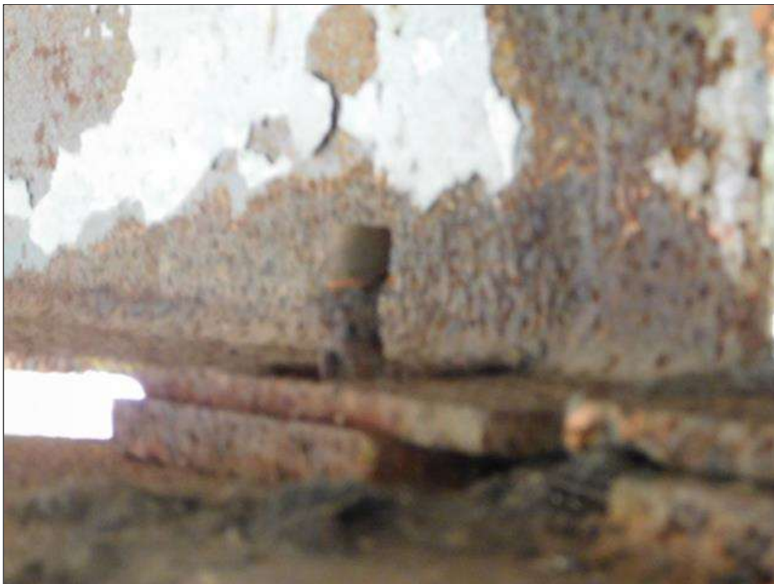
Span 5 Beam 4 - Near Bearing: BOTH ANCHOR BOLT NUTS MISSING. "PAR"
