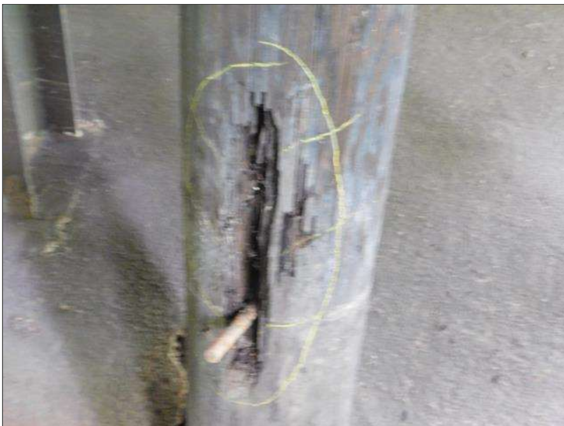
Bent 5 Pile 6: SOUTH AND NORTH FACE 4' BELOW CAP HAS AREAS OF DECAY UP TO 19" x 8" x 3" DEEP. "PAR"
