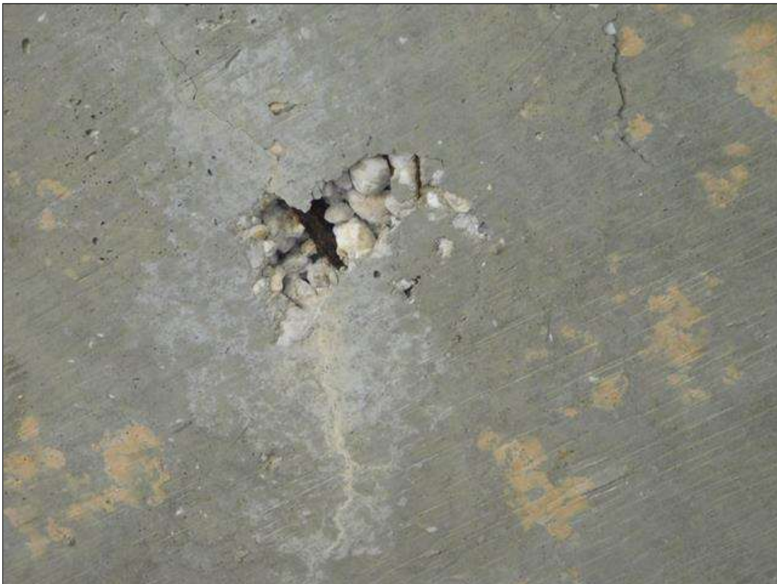
Span 5 Deck: 7" LONG X 7" WIDE X 1 1/2" DEEP SPALLED AREA WITH EXPOSED REINFORCEMENT IN THE UNDERSIDE OF THE DECK IN BAY 4, 7' FROM BENT 5
