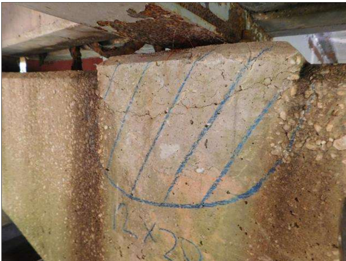
Bent 2 Cap 1: SOUTH FACE UNDER BEAM 2 HAS A 12" x 20" AREA THAT IS CRACKED AND DELAMINATED. SIMILAR AREA SOUTH FACE UNDER BEAM 3
