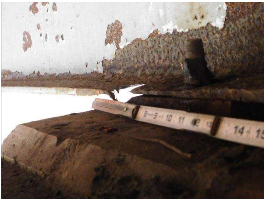
Span 3 Beam 3: BOTTOM FLANGE OVER BENT 2 HAS A AREA OF SECTION LOSS WITH DOWN TO KNIFE'S EDGE REMAINING. AREA IS: 12" LONG x FULL WIDTH. AREA ALSO HAS A 2" x 2 1/2" AREA OF 100% SECTION LOSS. "PAR"
