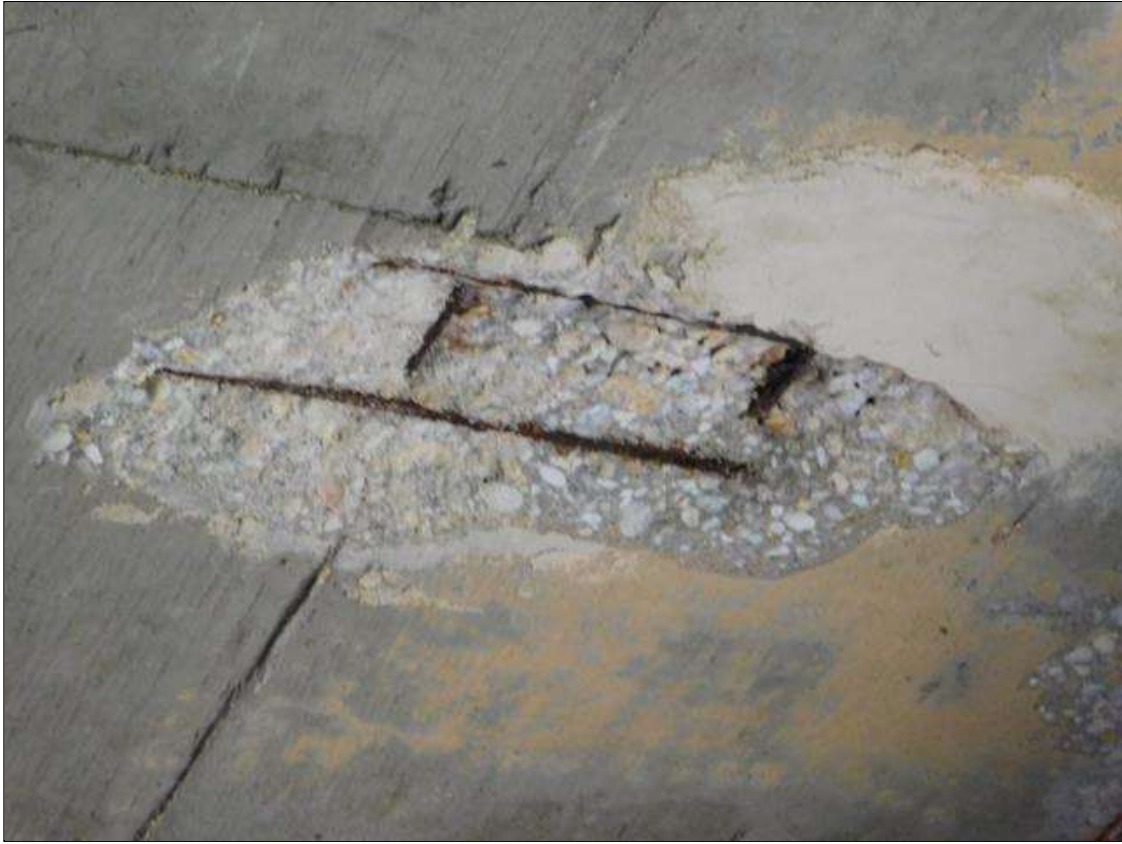
Span 6 Deck: 24" x 14" x 2" DEEP SPALL WITH EXPOSED REBAR. BOTTOM OF DECK BAY 4 NEAR MID-SPAN
