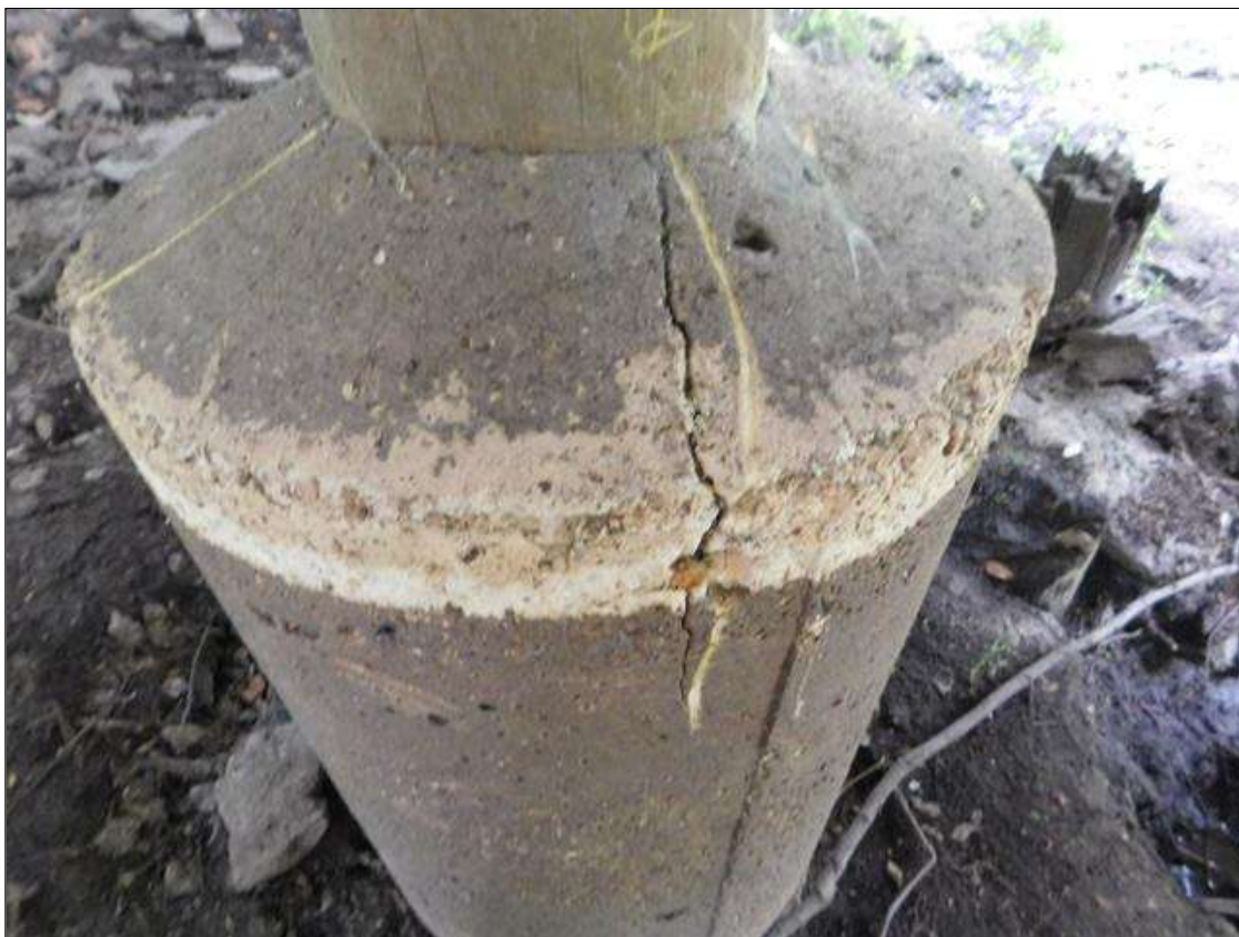
Bent 3 Pile 4: SCATTERED CHECKS UP TO 1/8" WIDE. CONCRETE ENCASEMENT HAS SCATTERED CRACKS UP TO 1/4" WIDE.
