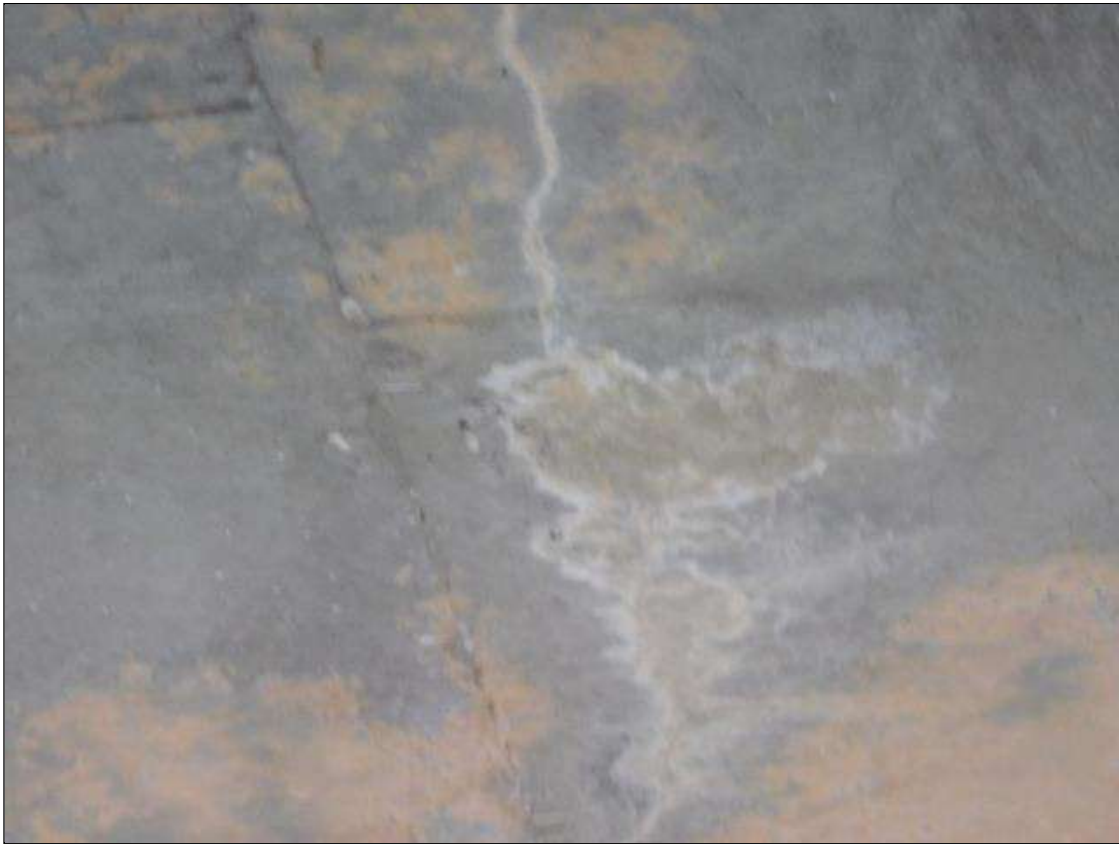
Span 5 Deck: INTERMITTENT FULL WIDTH X 1/32" WIDE TRANSVERSE CRACKS WITH EFFLORESCENCE IN THE UNDERSIDE OF THE DECK AT 1' TO 3' SPACING
