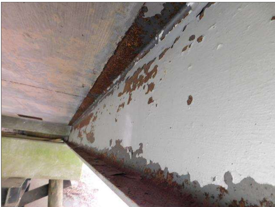
Span 1 Beam 1: SCATTERED AREAS OF RUST AND FLAKING IN BOTH FLANGES AND WEB
