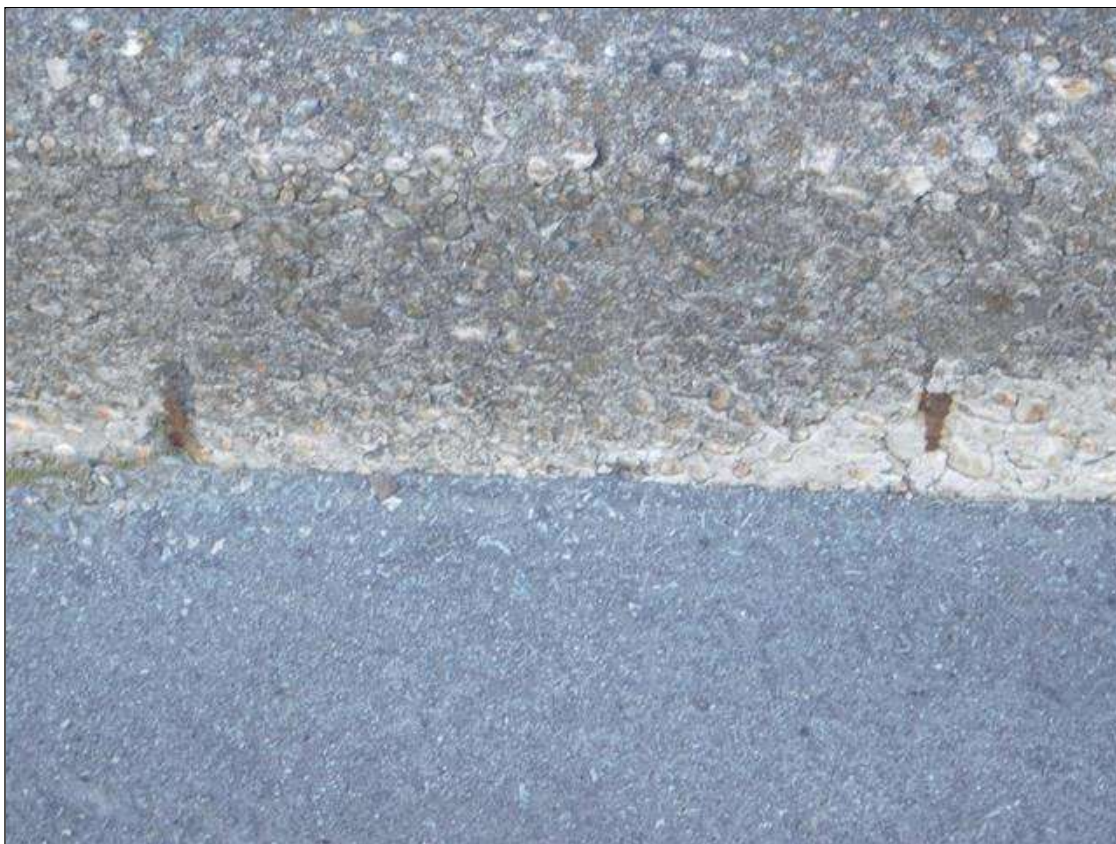
Span 2 Left Bridge Rail: (2) SPALLS IN FACE OF CURB WITH REBAR VISIBLE NEAR BENT 1. AREAS ARE 3" x 1" x 1/4" DEEP
