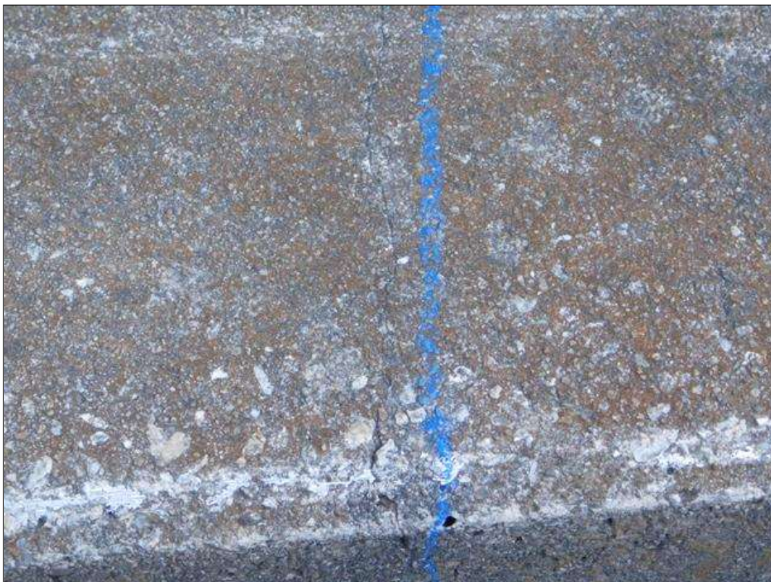
Span 6 Right Bridge Rail: 2'-9" LONG X 1/32" WIDE VERTICAL WRAP AROUND CRACK IN THE EAST CURB, 3' FROM BENT 5
