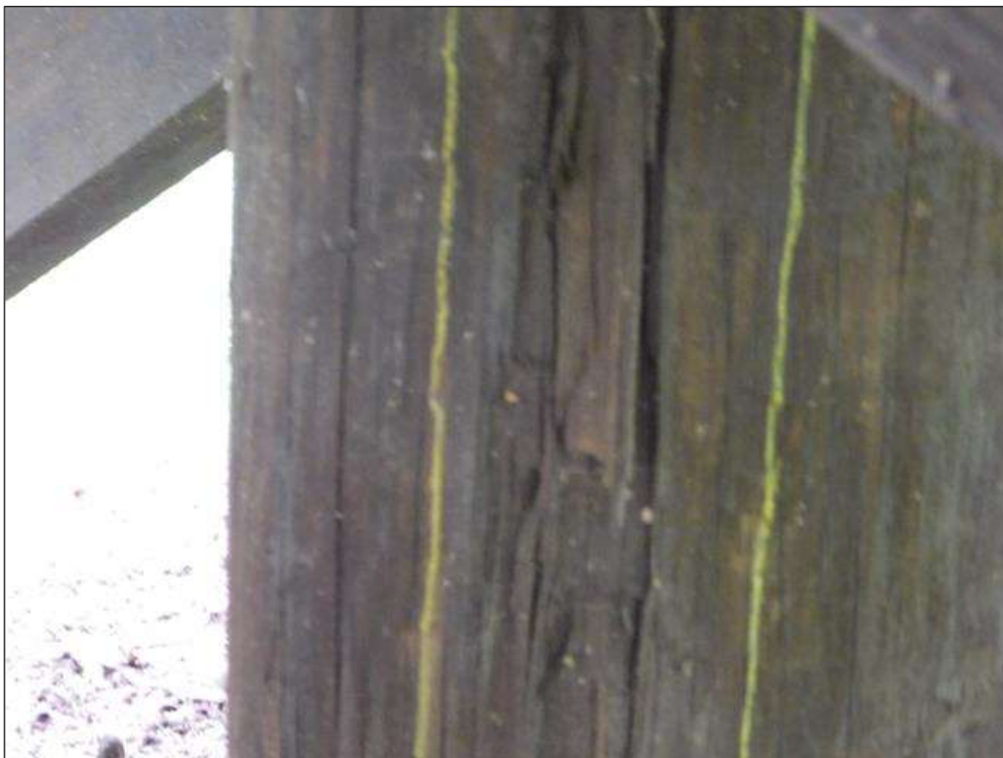
Bent 3 Pile 3: 36" TALL x 2" WIDE x 1/4" DEEP AREA OF DECAY ON SOUTH FACE BELOW CROSS-BRACE
