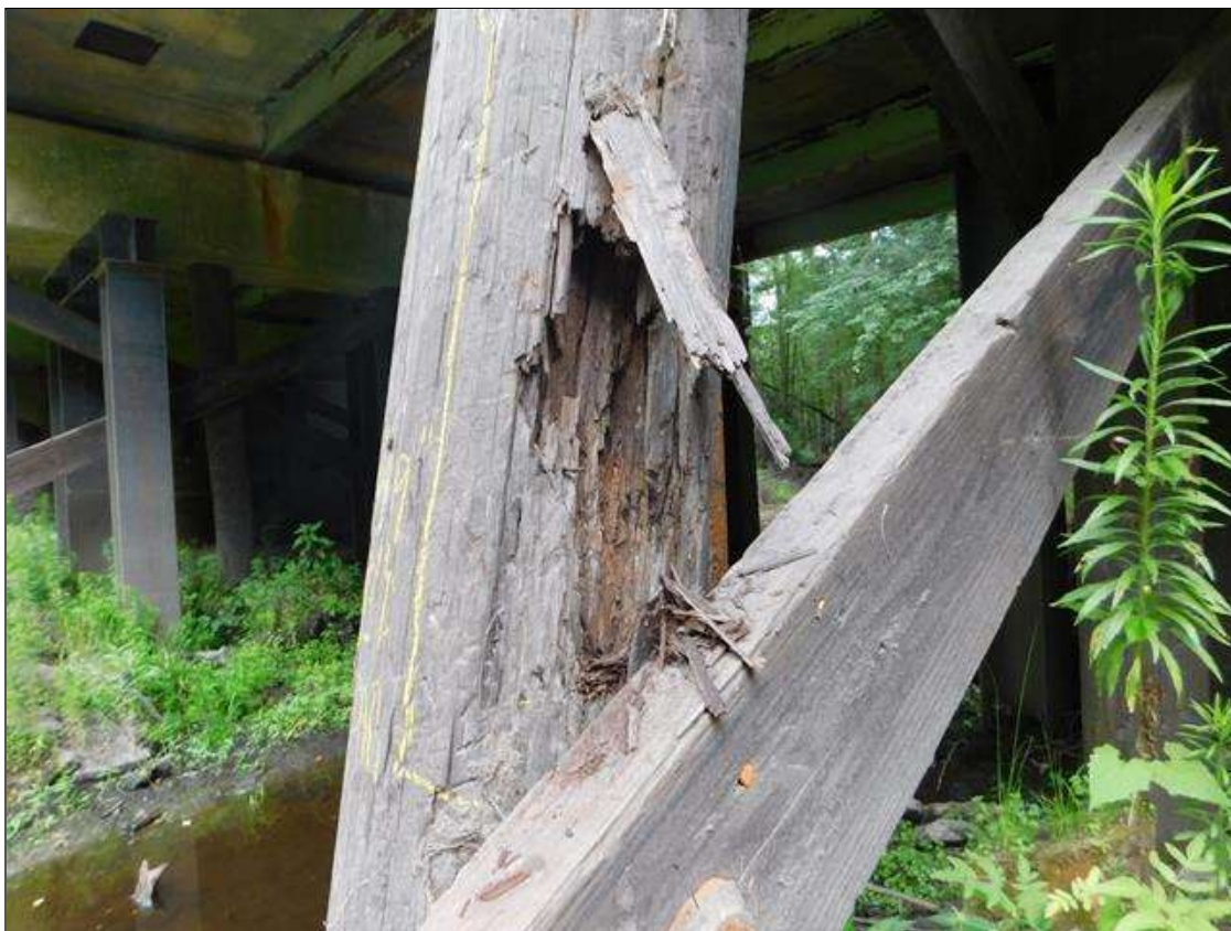
Bent 3 Pile 9: 4' x 9" x 3" DEEP AREA OF DECAY NORTH FACE OF LOWER CROSS-BRACE. "PAR"
