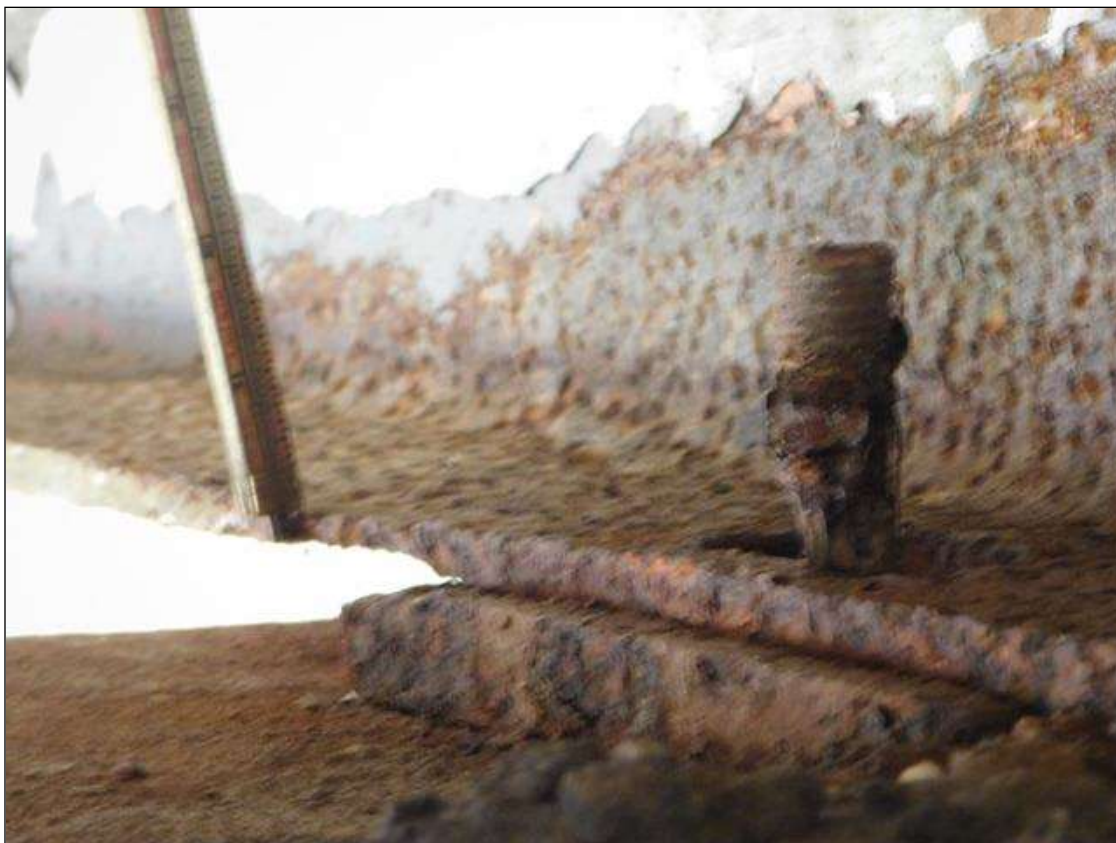
Span 5 Beam 3: BOTTOM FLANGE OVER BENT 4 HAS A AREA OF SECTION LOSS WITH 1/4" REMAINING. AREA IS: 10" LONG x FULL WIDTH. "PAR"
