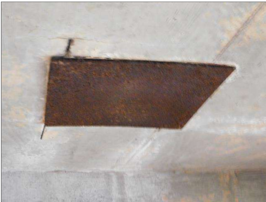
Span 1 Deck: METAL PLATE ATTACHED TO BOTTOM OF DECK IN BAYS 1, 3 AND 4 NEAR BENT 1
