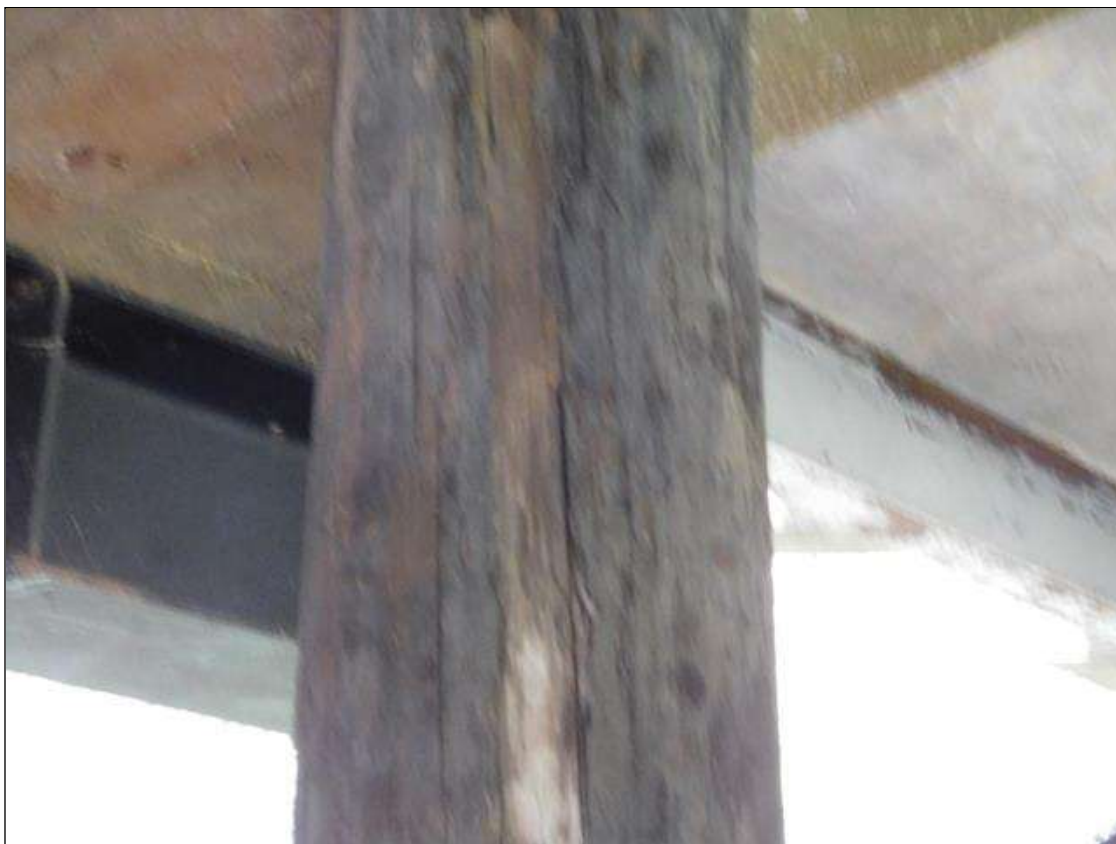
Bent 2 Pile 3: 30" TALL x 3" WIDE x 1/2" DEEP AREA OF DECAY IN SOUTH FACE AT TOP
