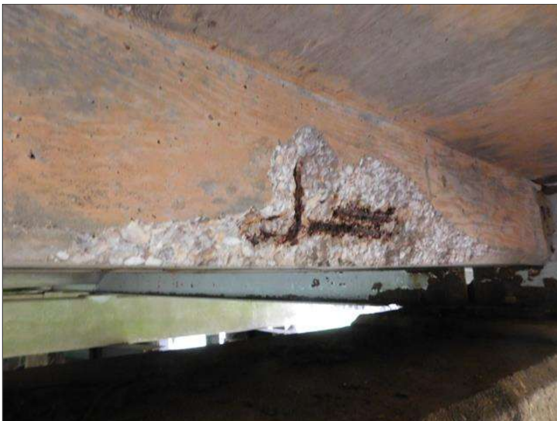
END DIAPHRAGM OVER BENT 2 IN BAY 2. HAS A 34" LONG x 8" HIGH x 2" DEEP SPALL WITH REBAR EXPOSED
