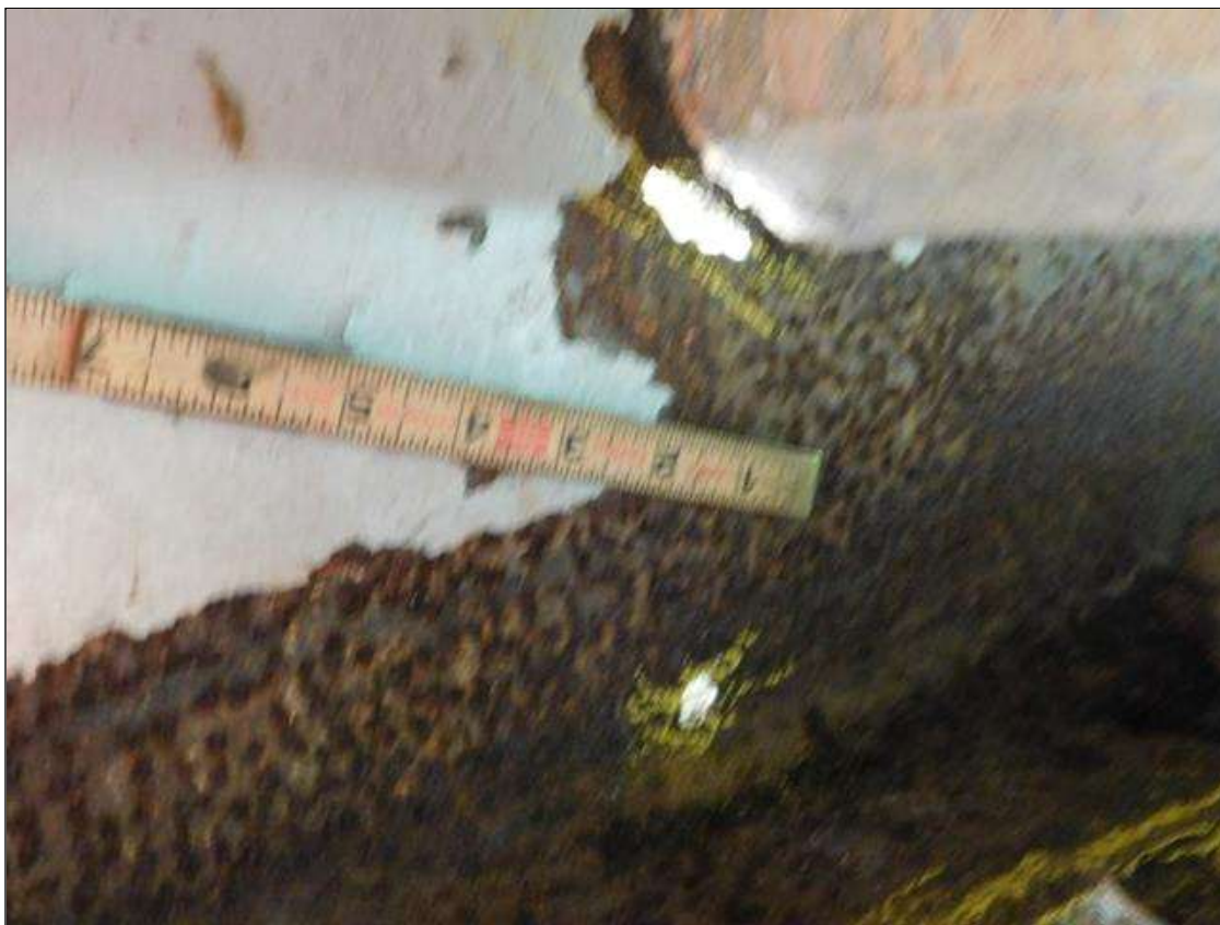
Span 1 Beam 1: WEB OVER BENT 2 HAS (2) AREAS OF 100% SECTION LOSS UP TO 1 1/2" x 1". "PAR" ISSUED
