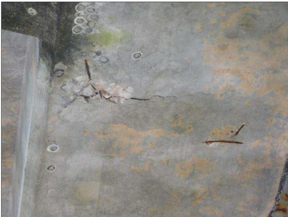
Span 4 Deck: 12" x 8" AREA OF DELAMINATION BOTTOM OF RIGHT OVERHANG 4' FROM BENT 3
