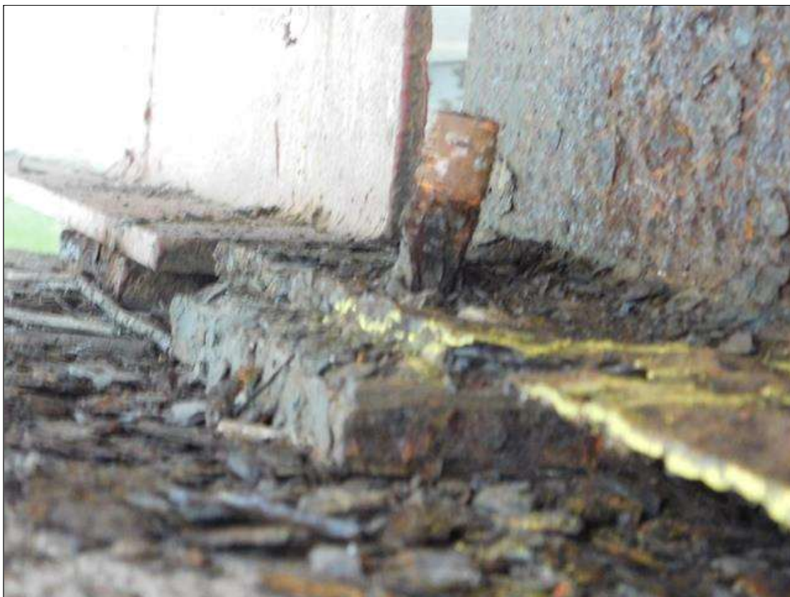
Span 1 Beam 1 - Far Bearing: SECTION LOSS WITH 3/4" REMAINING THRU-OUT BEARING AND LEFT ANCHOR BOLT NUT MISSING. "PAR" ISSUED
