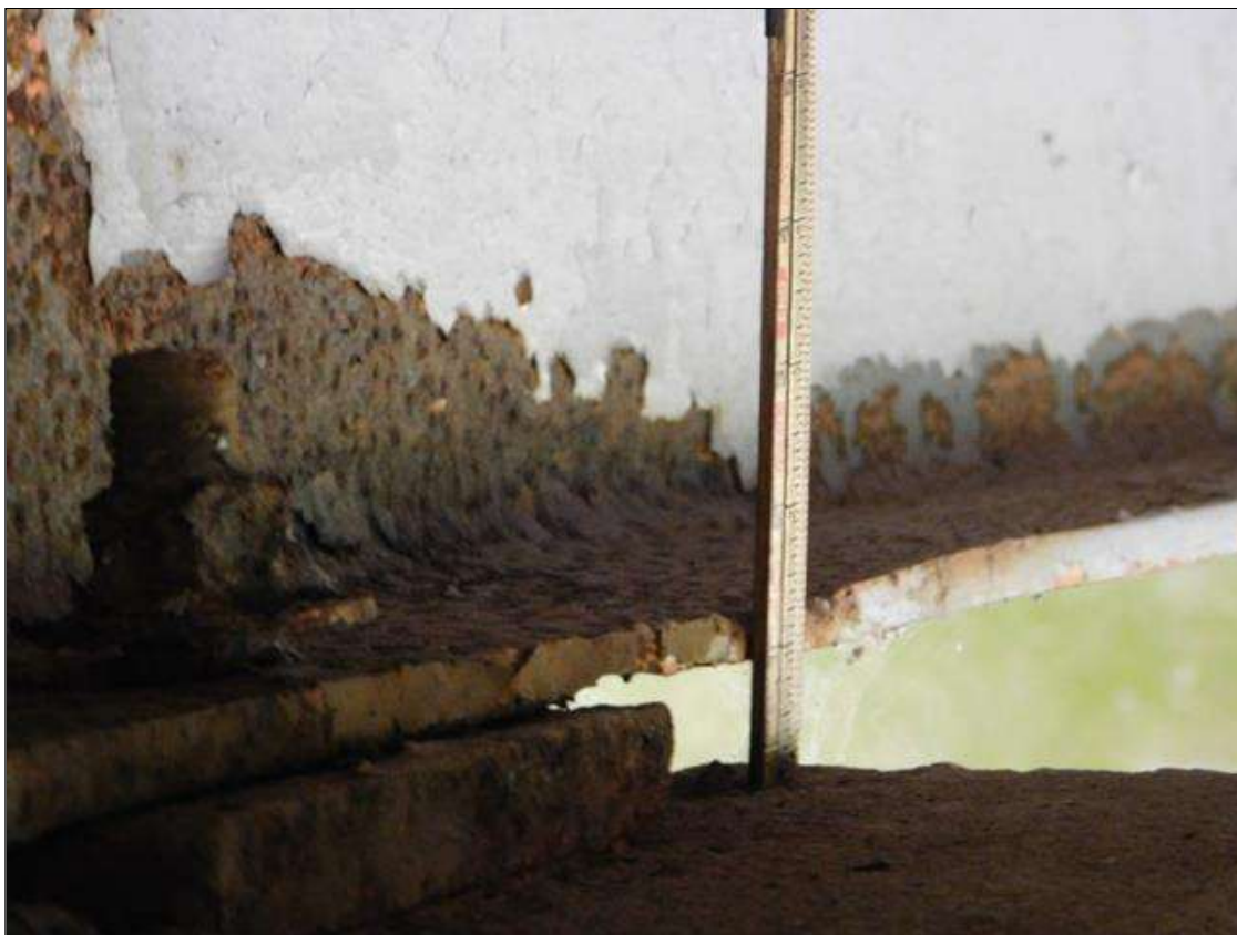
Span 3 Beam 2: RIGHT BOTTOM FLANGE OVER BENT 2 HAS A AREA OF SECTION LOSS WITH 1/4" REMAINING. AREA IS: 10" LONG x 3" WIDE. "PAR"
