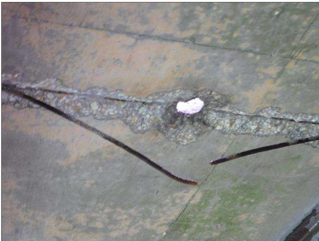
Span 5 Deck: 4' x 12" x 2" DEEP SPALL WITH BROKEN REBAR EXPOSED. BOTTOM OF DECK BAY 1 NEAR MID-SPAN. "PAR"
