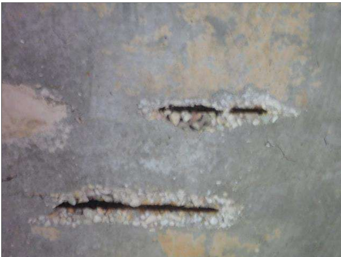
Span 5 Deck: (2) SPALLED AREAS WITH REBAR EXPOSED AND ADJACENT DELAMINATION. AREAS ARE UP TO 2' x 8" x 2" DEEP
