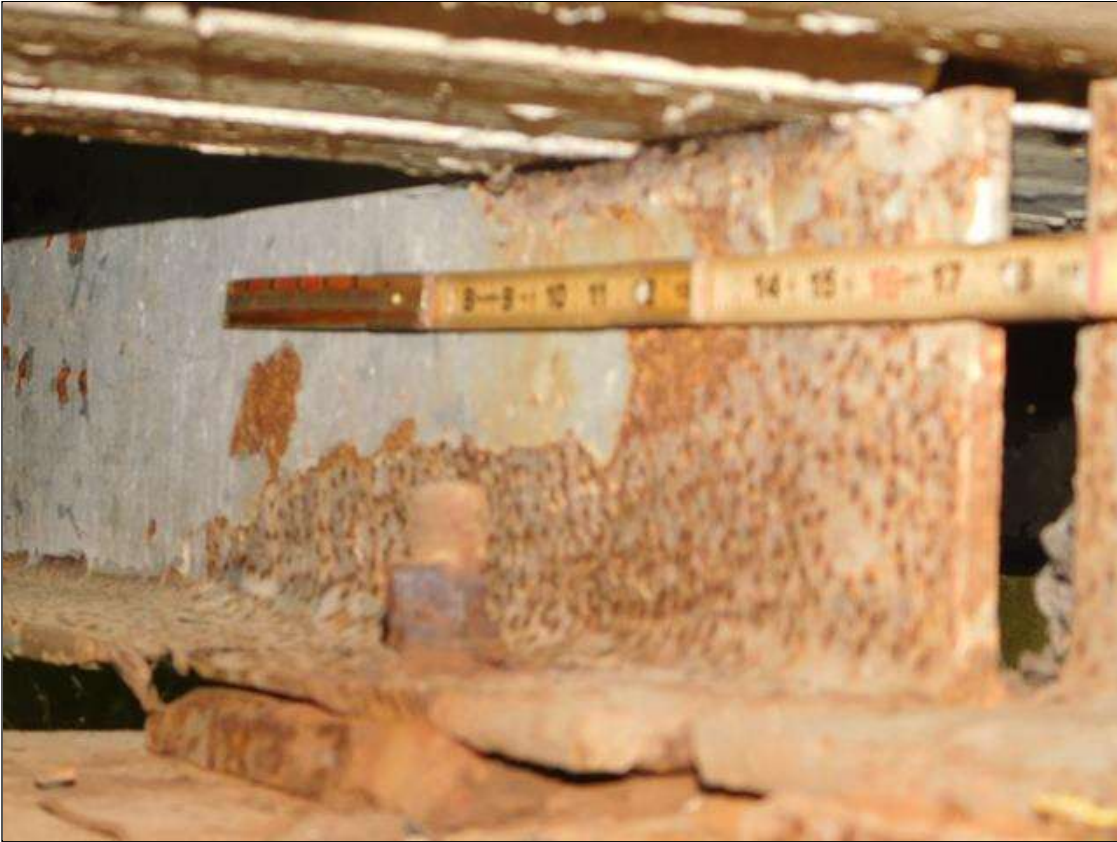
Span 3 Beam 3: WEB OVER BENT 2 HAS A AREA OF SECTION LOSS WITH 1/4" REMAINING. AREA IS: 18" LONG x UP TO 5" HIGH. "PAR"
