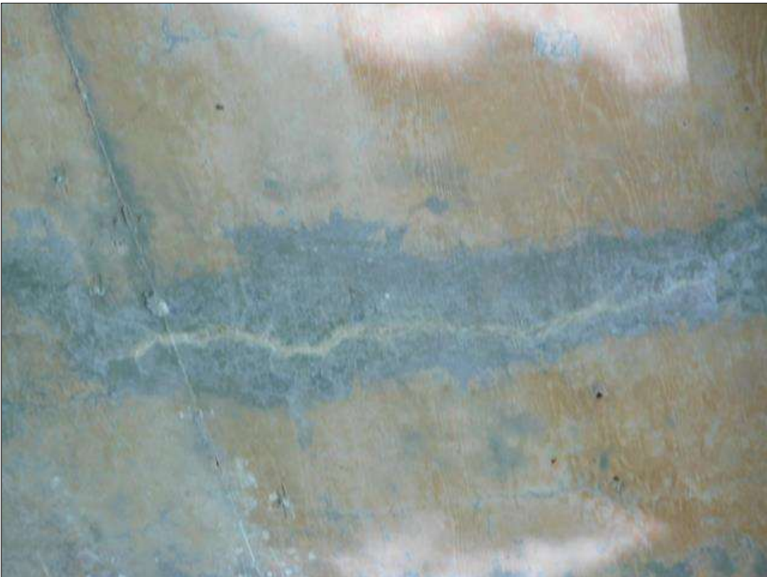
Span 3 Deck: SCATTERED HAIRLINE TRANSVERSE CRACKS UP TO FULL WIDTH WITH SOME EFFLO IN BOTTOM OF DECK
