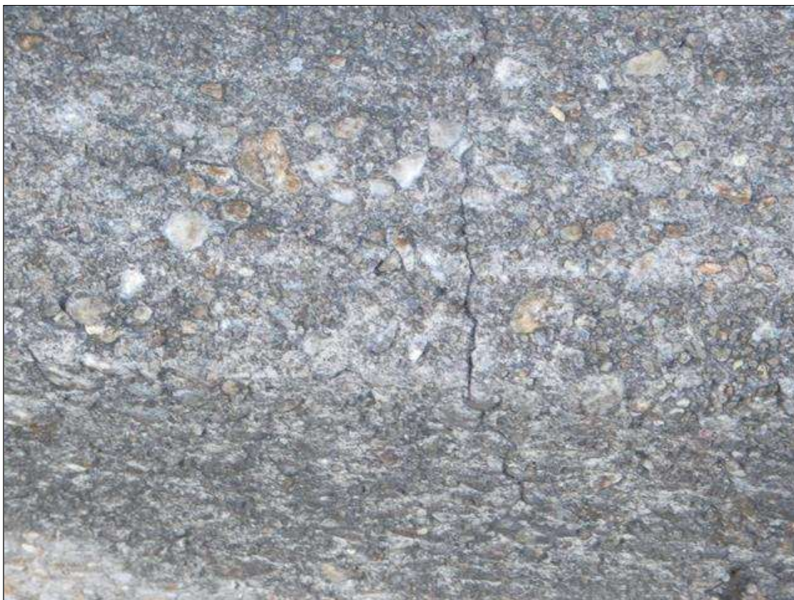
Span 1 Left Bridge Rail: SCATTERED HAIRLINE CRACKS IN FACE AND TOP OF CURB
