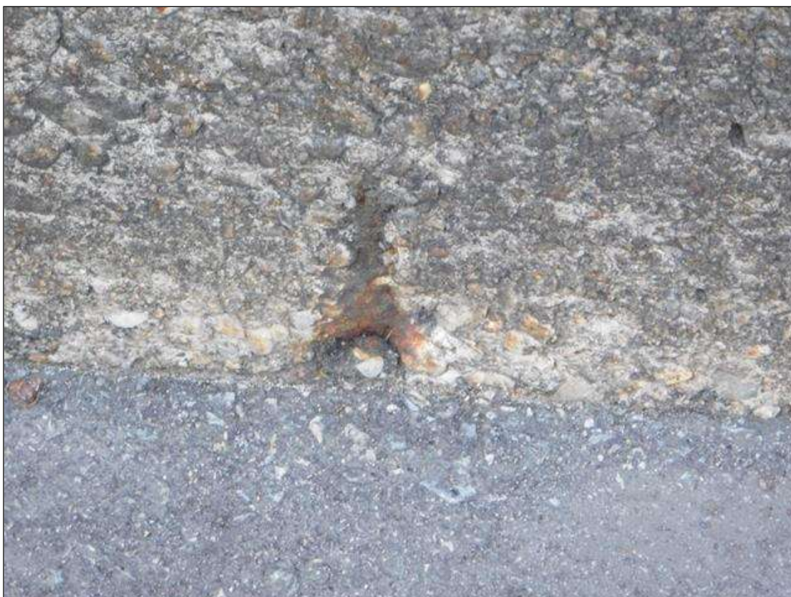
Span 1 Left Bridge Rail: 3" x 1" x 1/4" DEEP SPALL IN FACE OF CURB WITH RUST STAINS VISIBLE. 12' FROM END BENT 1
