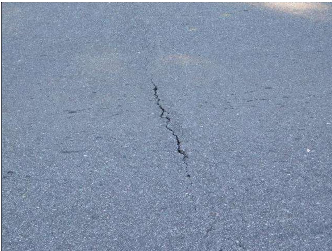
Span 2 Wearing Surface: SCATTERED TRANSVERSE CRACKS UP TO 1/8" WIDE OVER BENT 2
