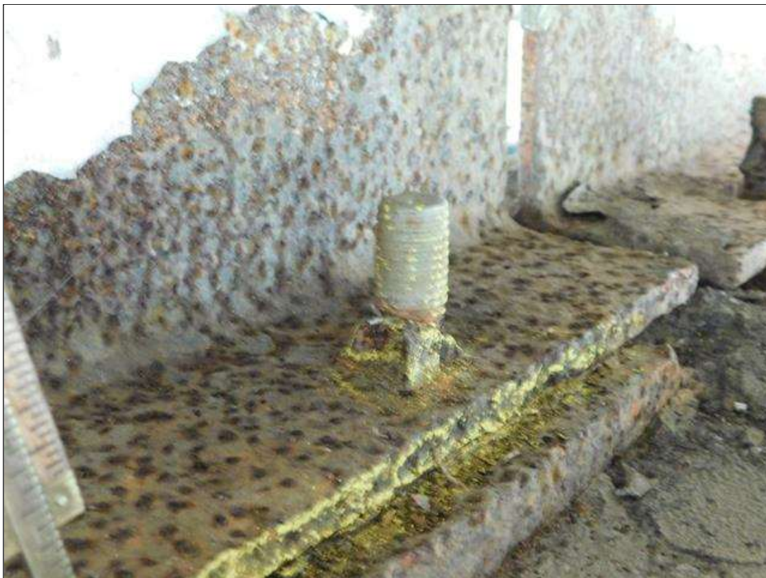
Span 3 Beam 3 - Far Bearing: RIGHT ANCHOR BOLT NUT MISSING. "PAR"
