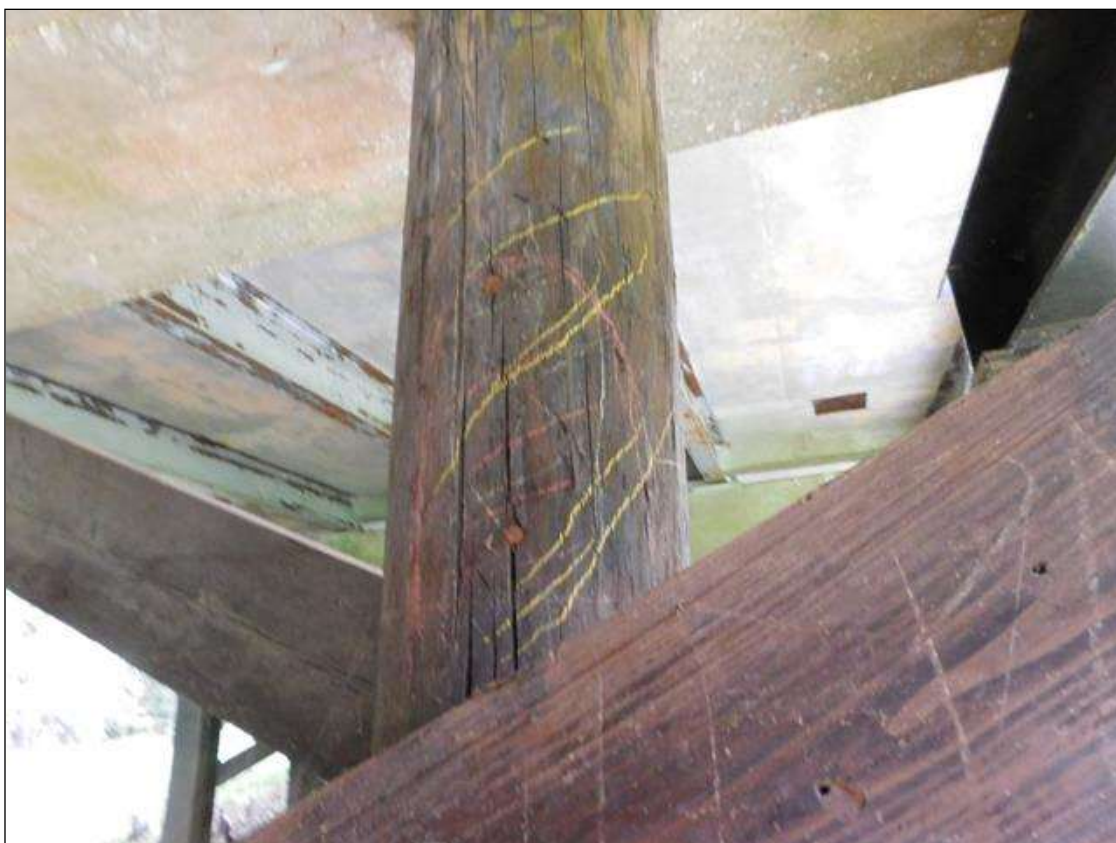
Bent 2 Pile 7: 5' HIGH x 1/2 CIRCUMFERENCE OF DELAMINATION WITH HOLLOW SOUND IN EAST FACE FROM TOP DOWN. "PAR" ISSUED
