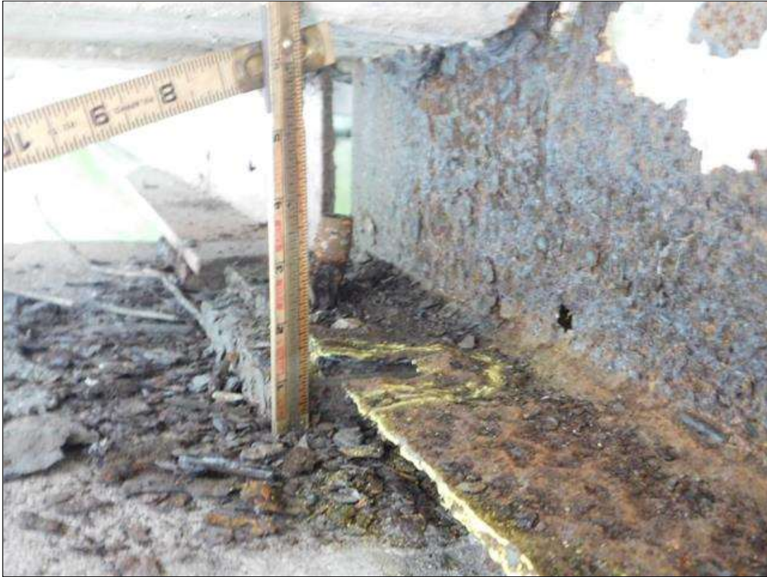
Span 1 Beam 1: LEFT BOTTOM FLANGE OVER BENT 2 HAS A AREA OF SECTION LOSS WITH DOWN TO KNIFE'S EDGE REMAINING. AREA IS: 18" LONG x 3" WIDE. AREA ALSO HAS 1 1/2" x 1 1/2" AREA OF 100% SECTION LOSS. "PAR" ISSUED
