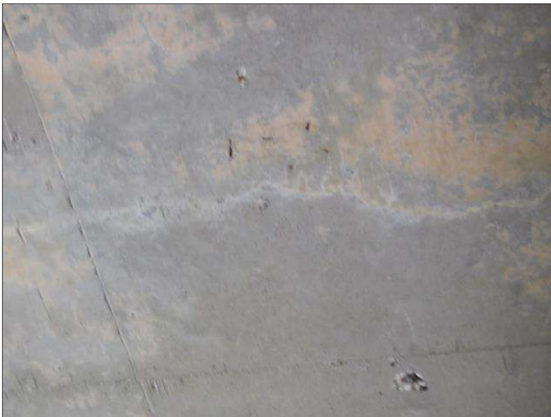
Span 6 Deck: SCATTERED HAIRLINE TRANSVERSE CRACKS UP TO FULL WIDTH IN BOTTOM OF DECK
