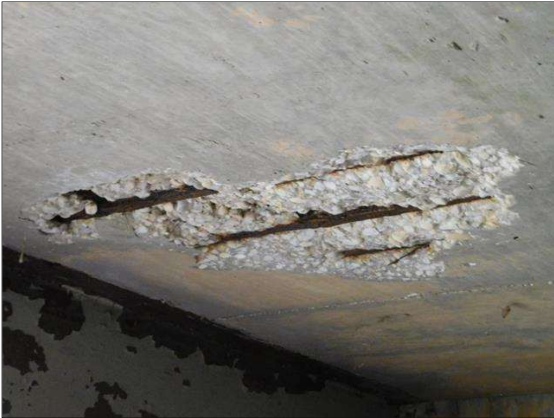
Span 1 Deck: 2' LONG X 2'-8" WIDE X 2" DEEP SPALLED AREA WITH EXPOSED REINFORCEMENT IN THE UNDERSIDE OF THE DECK IN BAY 4, 3' FROM END BENT 1
