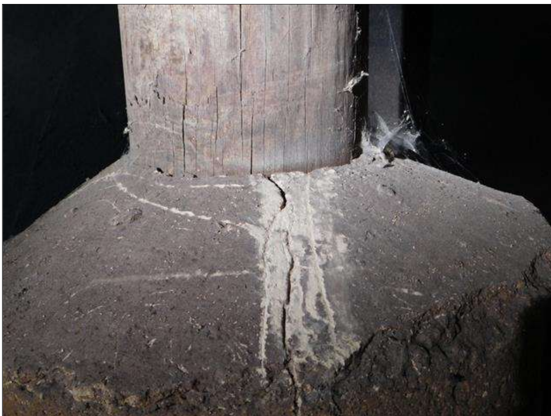
Bent 1 Pile 6: SCATTERED CHECKS UP TO 1/16" WIDE AND CONCRETE ENCASEMENT HAS SCATTERED CRACKS UP TO 1/8" WIDE
