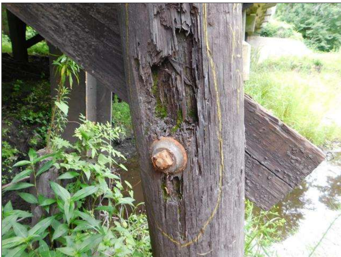
Bent 3 Pile 9: 23" x 6" x 2" DEEP AREA OF DECAY IN SOUTH FACE AND LOWER CROSS-BRACE. "PAR"
