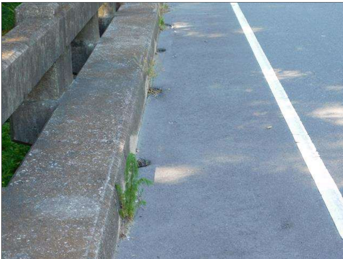
SCATTERED AREAS OF DEBRIS ADJACENT BOTH CURBS. TOTAL MAINTENANCE QUANTITY IS: 3388 Sq. Ft.
