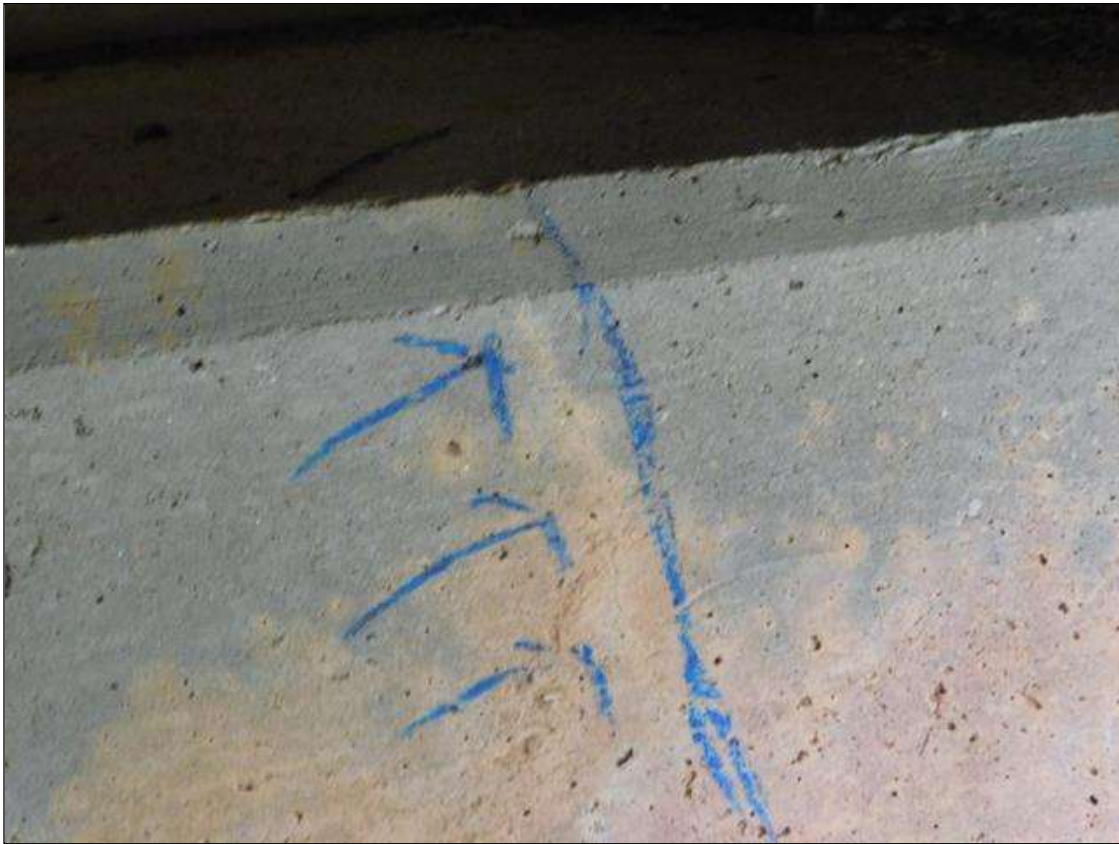
End Bent 2 Cap 1: SCATTERED HAIRLINE VERTICAL CRACKS
