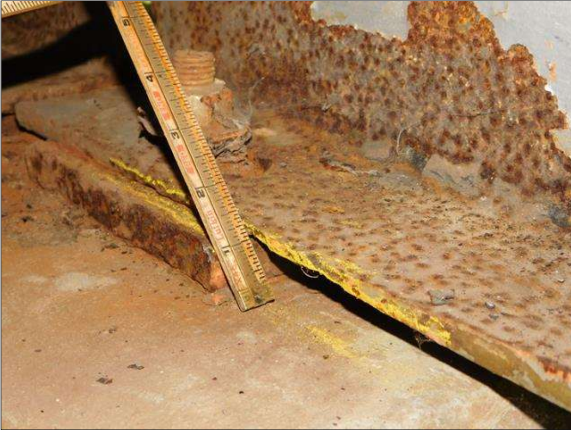
Span 1 Beam 3: BOTTOM FLANGE OVER BENT 2 HAS A AREA OF SECTION LOSS WITH DOWN TO 1/4" REMAINING. AREA IS: 10" LONG x FULL WIDTH. "PAR"
