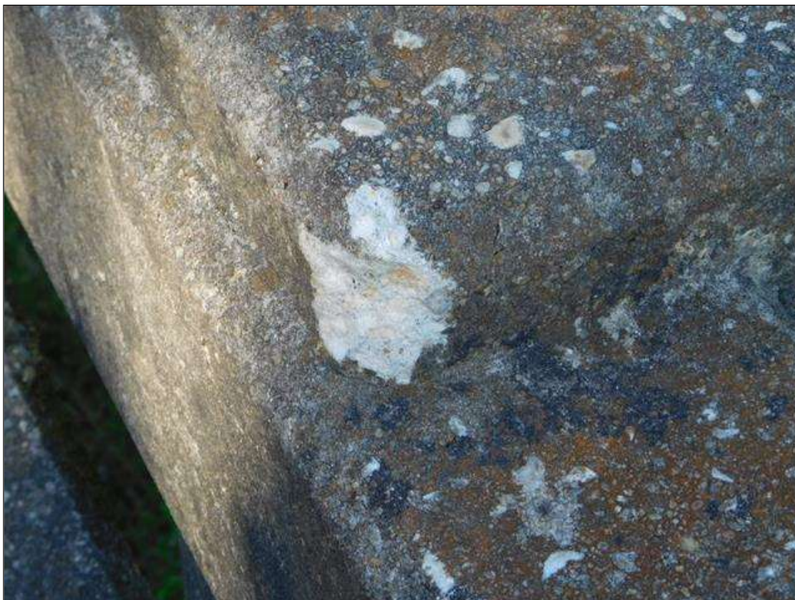
Span 2 Right Bridge Rail: SCATTERED SPALLS UP TO 4" x 3" x 1/2" DEEP IN FACE OF RAIL AND POST
