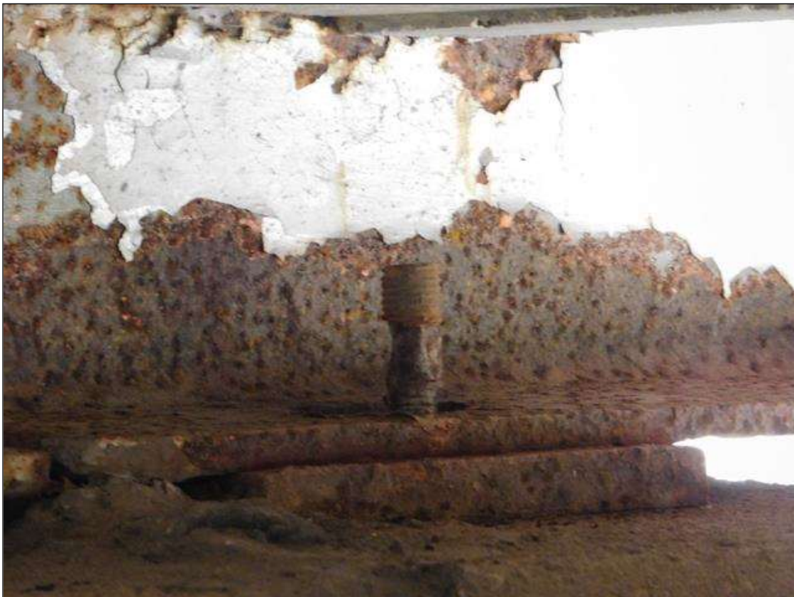
Span 5 Beam 2 - Near Bearing: RIGHT ANCHOR BOLT NUT MISSING. "PAR"
