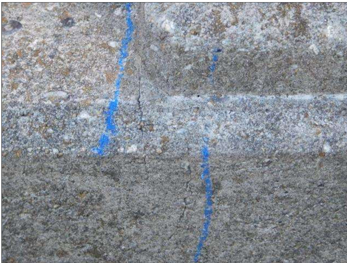
Span 6 Left Bridge Rail: SCATTERED HAIRLINE CRACKS IN RAIL AND CURB NEAR END BENT 2
