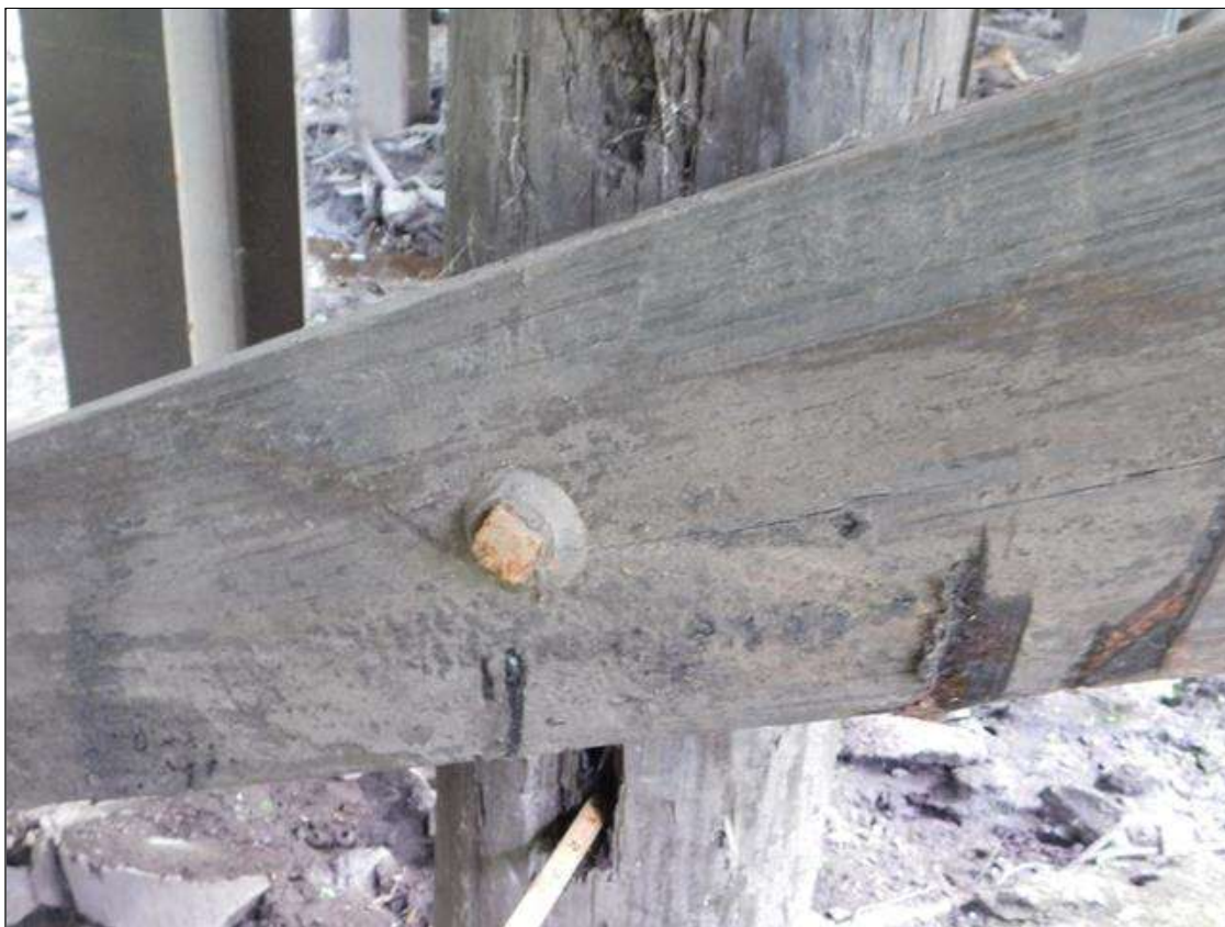
Bent 2 Pile 6: 18" TALL x 3" WIDE x 1 1/2" DEEP AREA OF DECAY IN SOUTH FACE AT LOWER CROSS-BRACE.
