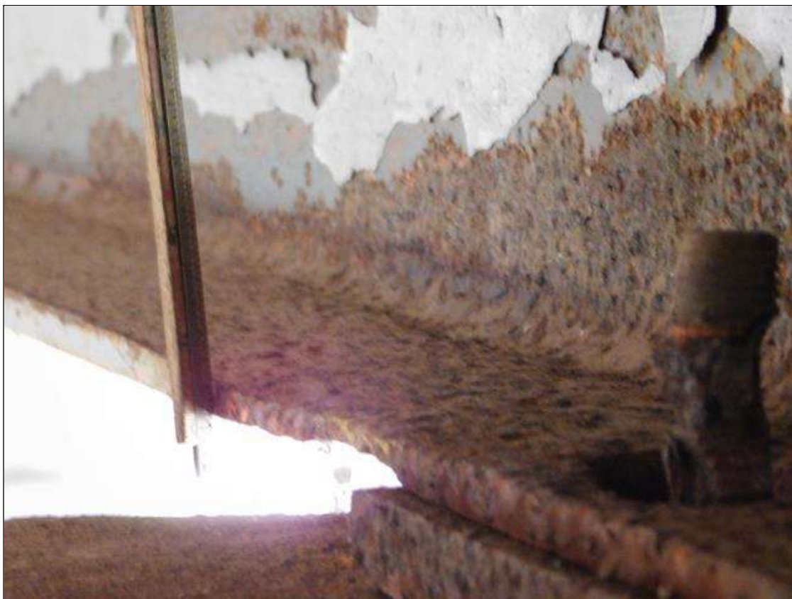
Span 5 Beam 4: BOTTOM FLANGE OVER BENT 4 HAS A AREA OF SECTION LOSS WITH DOWN TO 1/8" REMAINING. AREA IS UP TO 20" LONG x FULL WIDTH. "PAR"
