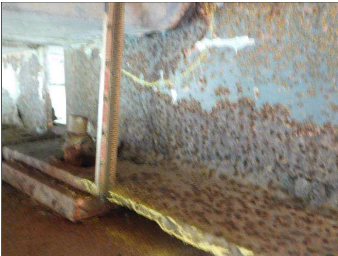
Span 1 Beam 2: BOTTOM FLANGE AND WEB OVER BENT 2 HAS AREAS OF SECTION LOSS. WEB AREA IS: 6" LONG x 1" TALL WITH 1/4" REMAINING. BOTTOM FLANGE AREA IS: 12" LONG x FULL WIDTH WITH DOWN TO 1/4" REMAINING. "PAR"
