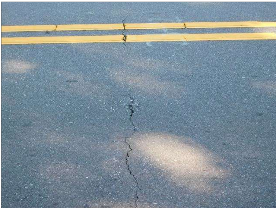
Span 1 Wearing Surface: SCATTERED TRANSVERSE CRACKS UP TO 1/8" WIDE OVER END BENT 1
