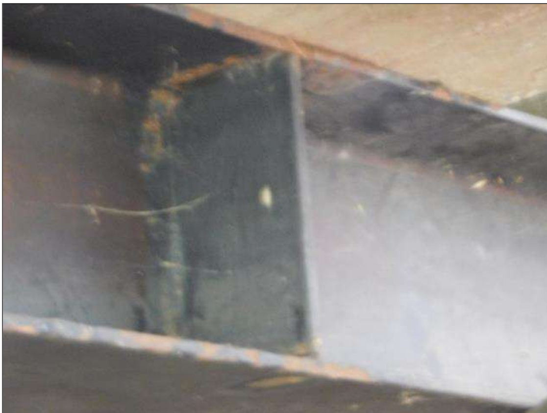
Bent 1 Pile 2 (Crutch Bent): SCATTERED AREAS OF SURFACE RUST (6 FT.)
