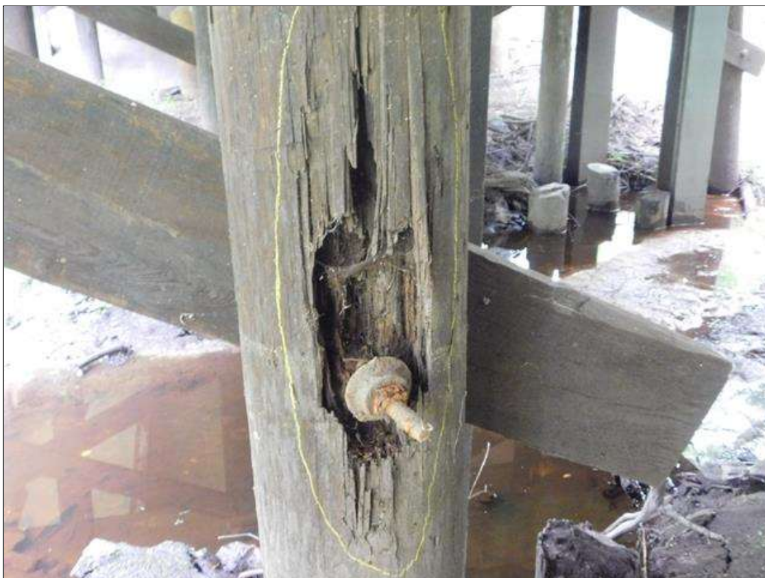
Bent 3 Pile 6: 28" x 5" x 4" DEEP AREA OF DECAY ON NORTH FACE OF LOWER CROSS-BRACE. "PAR"
