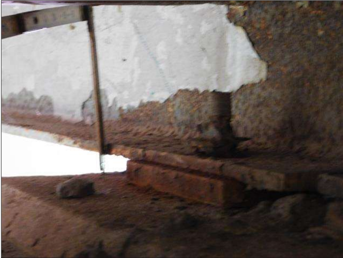
Span 3 Beam 4: BOTTOM FLANGE OVER BENT 2. HAS A AREA OF SECTION LOSS WITH 5/16" REMAINING. AREA IS: 12" LONG x FULL WIDTH. "PAR" ISSUED
