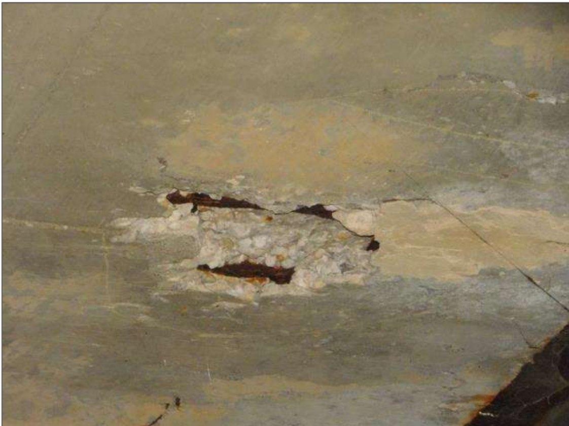
Span 6 Deck: 16" DIAMETER x 2" DEEP SPALL WITH EXPOSED REBAR. BOTTOM OF DECK BAY 4 AT END BENT
