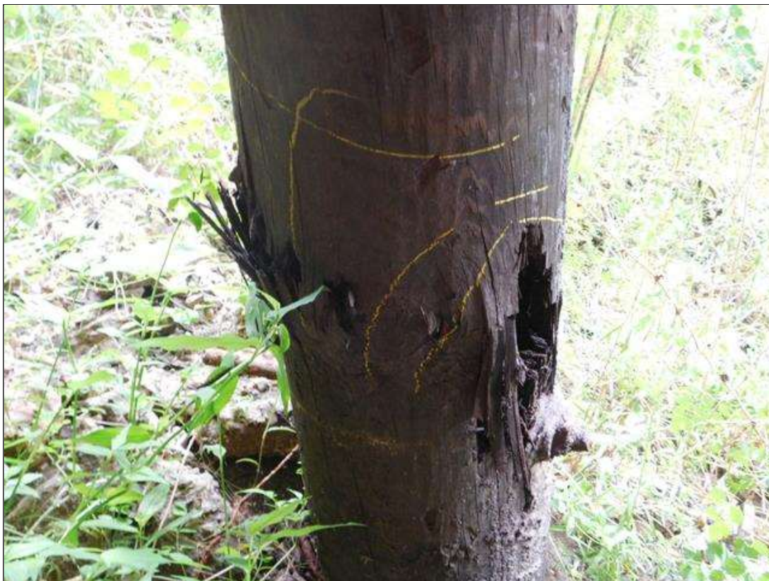
Bent 5 Pile 9: 12" TALL x FULL CIRCUMFERENCE x 2" DEEP AREA OF DECAY. 16" ABOVE GROUNDLINE. "PAR"
