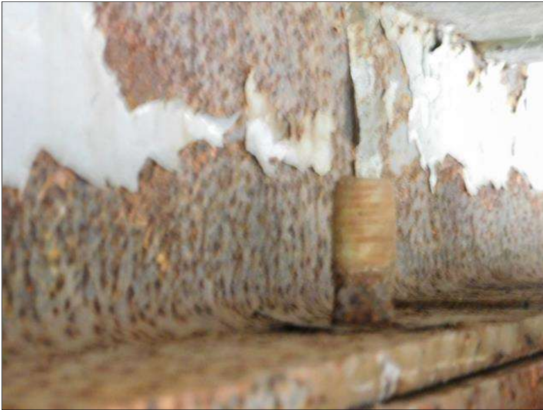
Span 3 Beam 2 - Far Bearing: ANCHOR BOLT NUT MISSING ON BOTH SIDES. "PAR"
