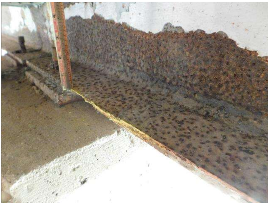
Span 3 Beam 4: BOTTOM FLANGE OVER BENT 4 HAS A AREA OF SECTION LOSS WITH 1/8" REMAINING. AREA IS: 10" LONG x FULL WIDTH. "PAR"
