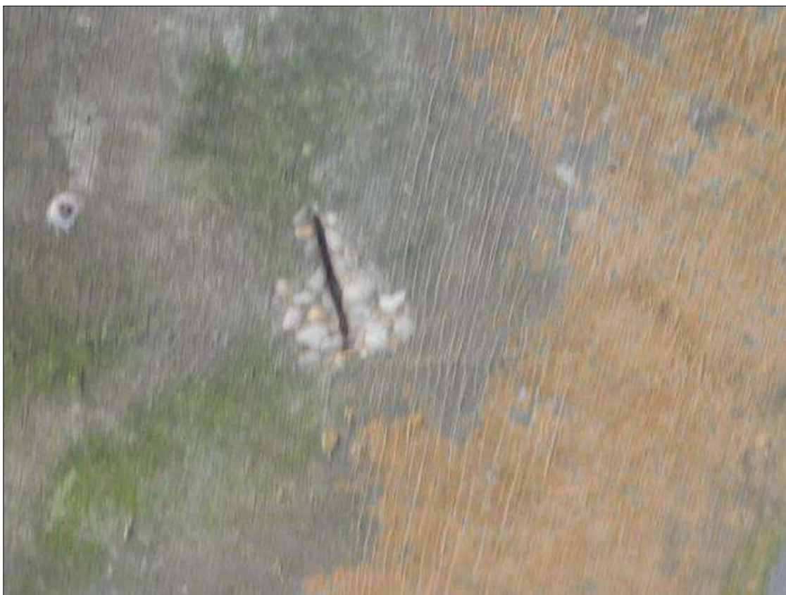
Span 2 Deck: 6" x 3" x 1/4" DEEP SPALL WITH REBAR VISIBLE IN BOTTOM OF LEFT OVERHANG. 6' FROM BENT
