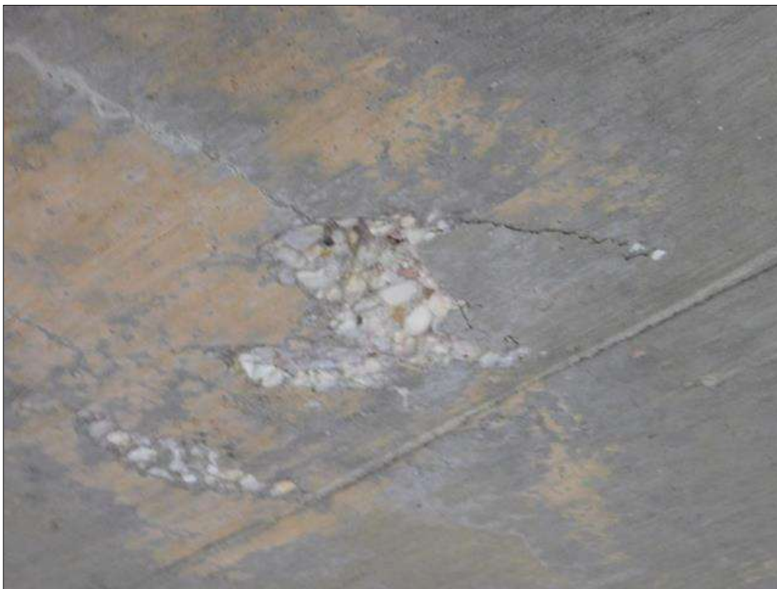
Span 6 Deck: 20" x 16" AREA THAT IS CRACKED AND DELAMINATED WITH (2) SPALLS UP TO 10" x 8" x 1" DEEP. BOTTOM OF DECK IN BAY 1 NEAR MID-SPAN
