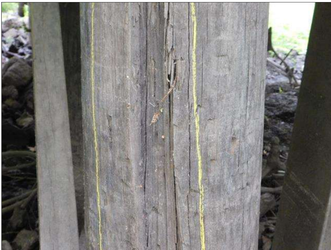
Bent 4 Pile 1: 30" x 2 1/2" x 1 1/2" DEEP AREA OF DECAY IN WEST FACE 2' BELOW CAP
