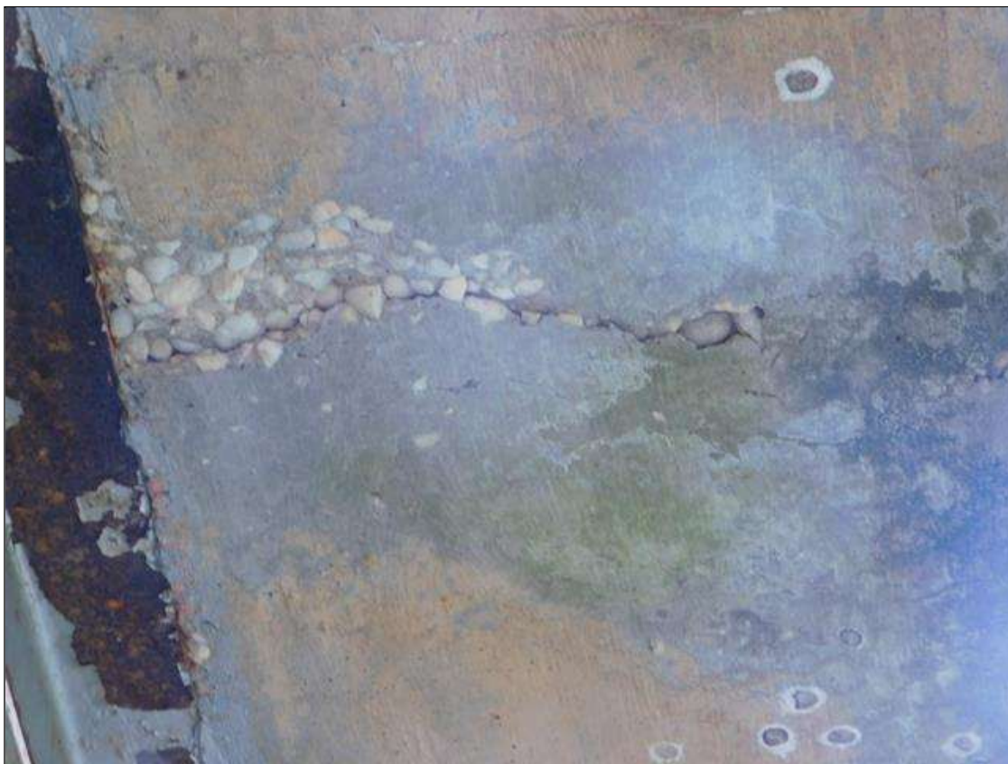
Span 2 Deck: 3' WIDE x 18" LONG CRACKED AND DELAMINATED AREA IN BOTTOM OF RIGHT OVERHANG. 5' FROM BENT 2
