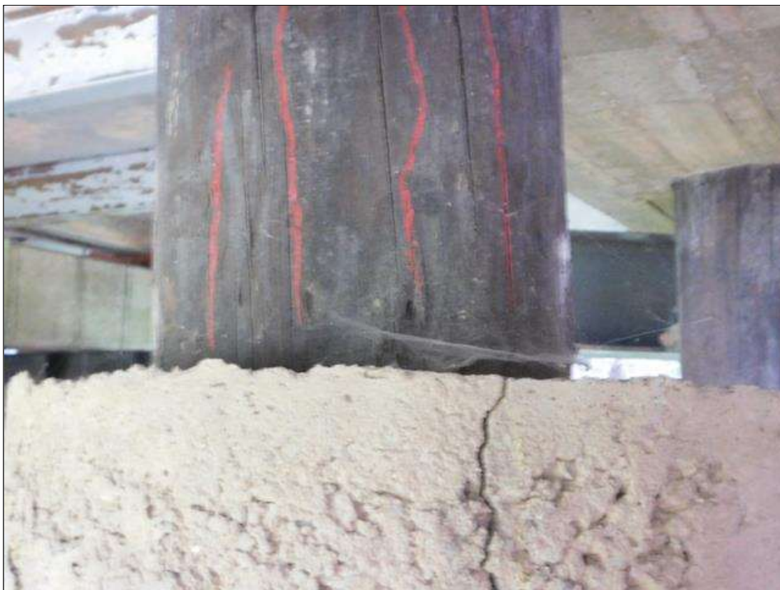
Bent 5 Pile 7: SCATTERED CHECKS UP TO 1/8" WIDE WITH A CONCRETE ENCASEMENT ON EAST FACE THAT HAS A FULL HEIGHT x 1/4" WIDE CRACK
