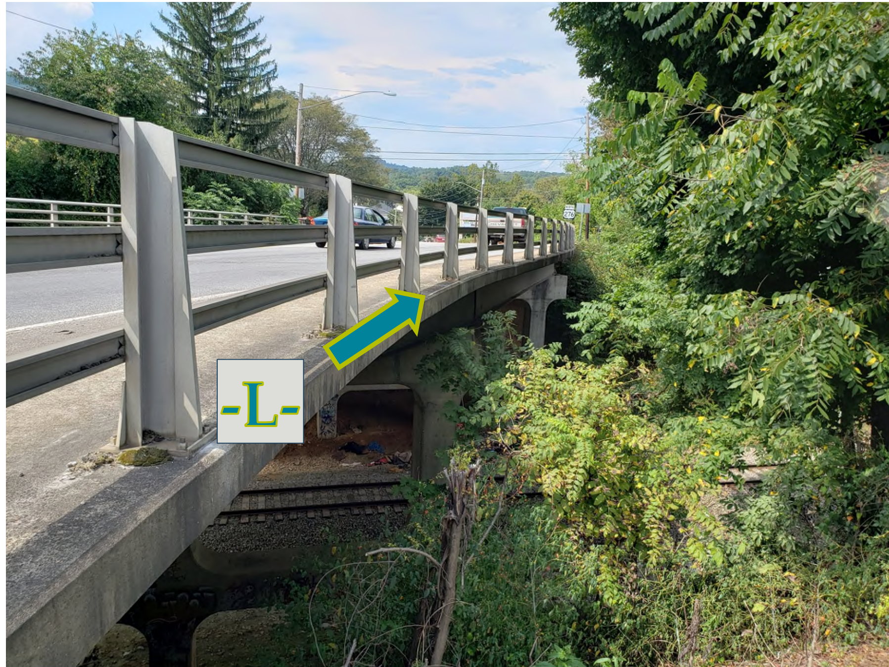
Bridge No. 184 on -L- (US 276) over Blue Ridge Southern Railroad Looking North Toward End Bent 2
