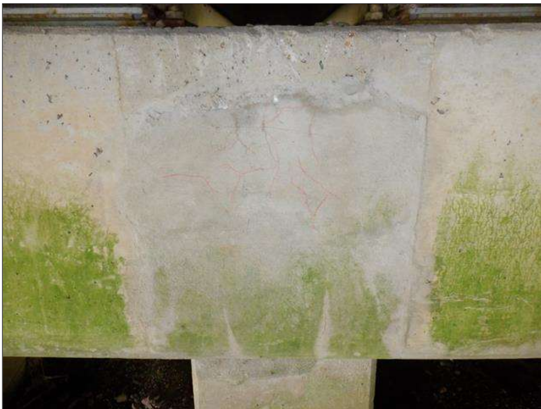
Bent 1 Cap 1: 3 FEET X UP TO 3 FEET CRACKED PATCHED AREA WITH HAIRLINE MAP CRACKING ON NORTH FACE BETWEEN BEAMS 4 AND 5.
