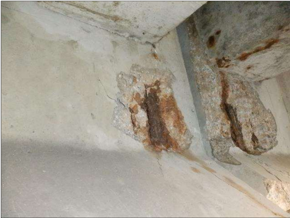
Span 2 Beam 7: (3) UP TO 7.5 INCHES X 9 INCHES X 1 INCHES SPALLS WITH EXPOSED REINFORCING ON EAST AND WEST FACES OF WEB AND CHAMFER AT BENT 2.
