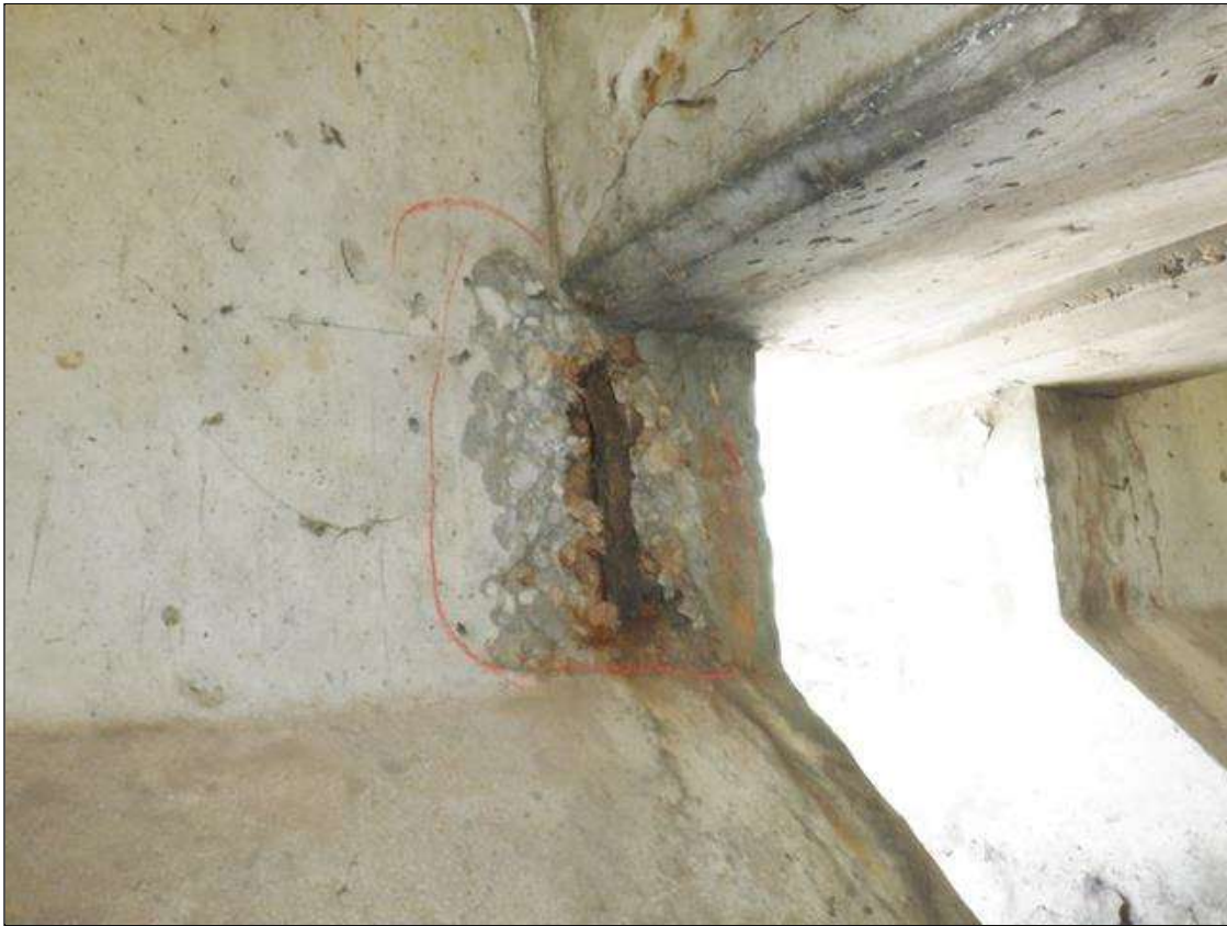
Span 1 Beam 1: 6 INCHES X UP TO 8 INCHES X 1 INCHES SPALL WITH EXPOSED REINFORCING ON EAST FACE AT BENT 1.
