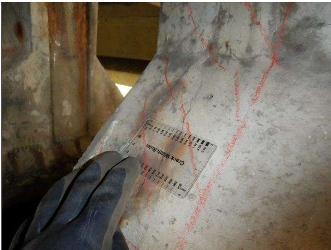
Span 2 Beam 3: (PAR) 7 INCHES X UP TO 0.016 INCHES VERTICAL CRACK WITH RUST STAINING AND ADJACENT 7 INCHES X 14 INCHES DELAMINATION AND HAIRLINE CRACKING IN THE EAST FACE OF THE WEB AND CHAMFER AT BENT 1.
