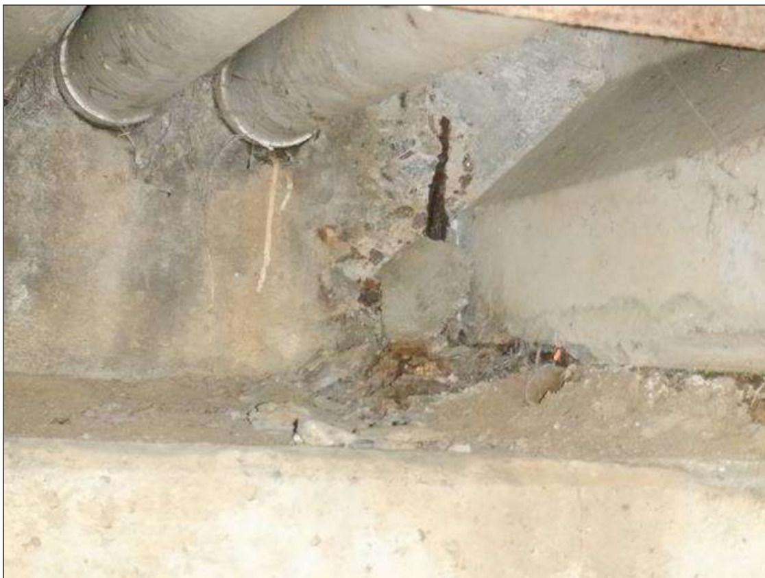
End Bent 2 Abutment: 6 INCHES X UP TO 12 INCHES X 1 INCHES SPALL WITH EXPOSED REINFORCING ON SOUTH FACE BETWEEN BEAMS 7 AND 8, NEAR BEAM 8.
