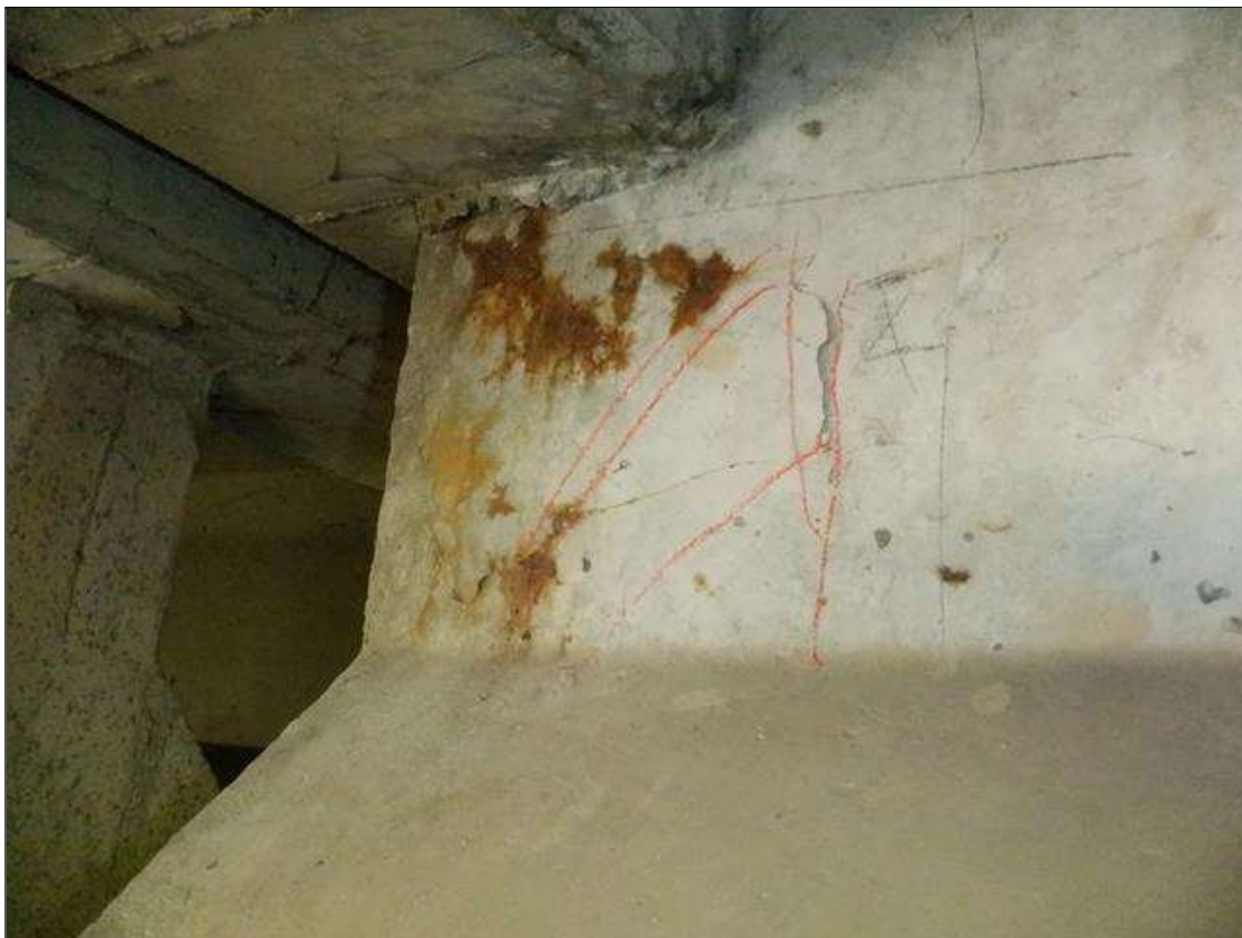
Span 1 Beam 4: 10 INCHES X UP TO 6 INCHES DELAMINATION WITH HAIRLINE MAP CRACKING AND RUST STAINING ON WEST FACE AT BENT 1.
