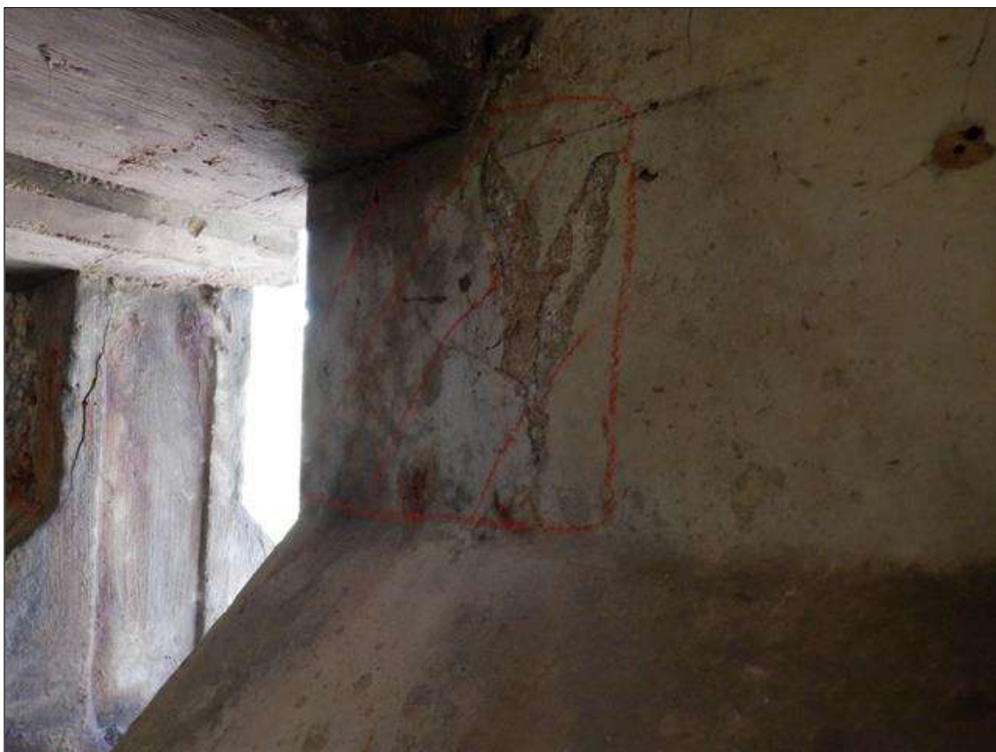
Span 2 Beam 1: 6 INCHES X UP TO 6 INCHES DELAMINATION/SURFACE SPALL WITH HAIRLINE MAP CRACKING AND RUST STAINING ON EAST FACE AT BENT 1.
