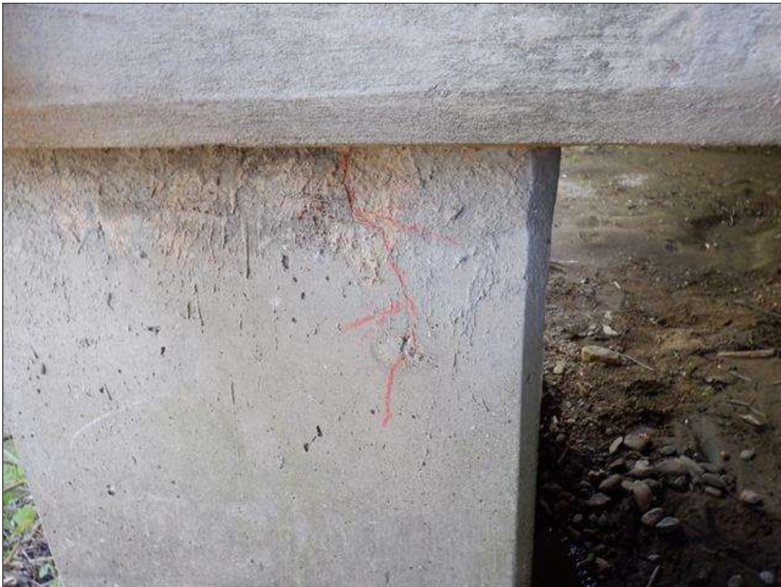
Bent 1 Pile 8: 12 INCHES X UP TO 1/64 INCHES VERTICAL CRACK ON NORTH FACE AT BOTTOM OF CAP.
