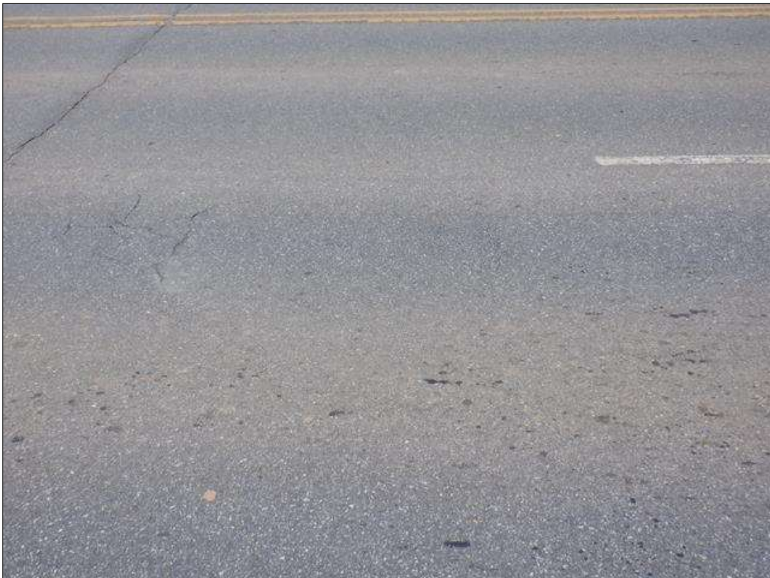
Span 1 Wearing Surface: 20 SQUARE FEET OF UP TO 1/16 INCHES MAP CRACKING AT RANDOM THROUGHOUT.
