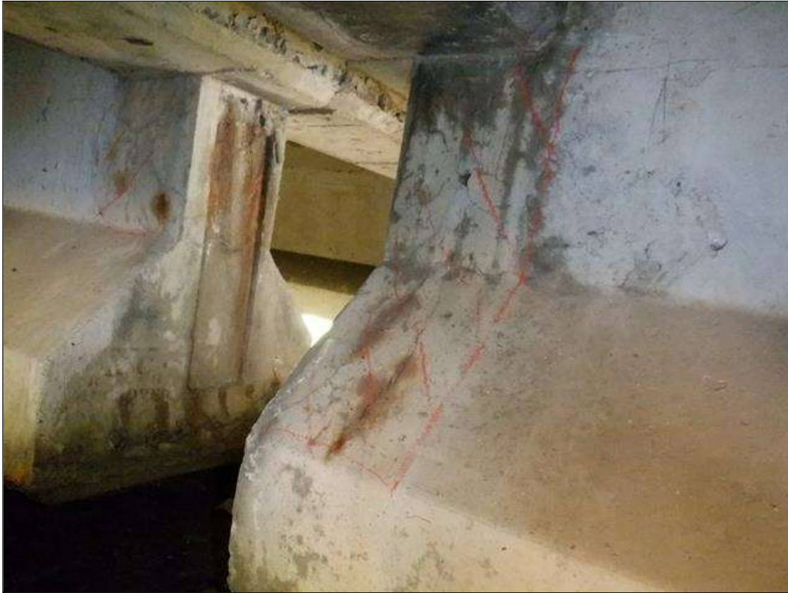
Span 2 Beam 3: (PAR) 7 INCHES X UP TO 0.016 INCHES VERTICAL CRACK WITH RUST STAINING AND ADJACENT 7 INCHES X 14 INCHES DELAMINATION AND HAIRLINE CRACKING IN THE EAST FACE OF THE WEB AND CHAMFER AT BENT 1.
