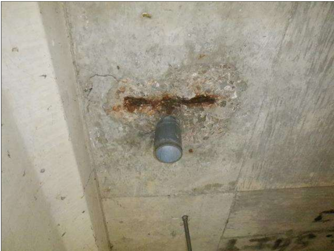
Span 2 Deck: 16 INCHES X UP TO 10 INCHES X 1 INCHES SPALL WITH EXPOSED REINFORCING ON DECK UNDERSIDE AROUND FIRST DRAIN BETWEEN BEAMS 7 AND 8 MEASURED FROM BENT 1.
