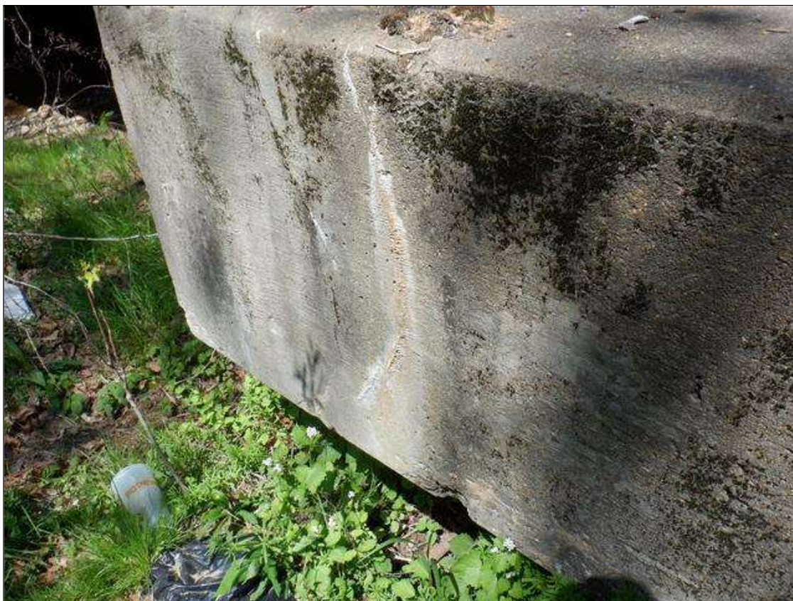
Bent 1 Cap 1: 30 INCHES X UP TO 1/64 INCHES VERTICAL CRACKS WITH EFFLORESCENCE AND HEAVY BUILDUP ON WEST FACE.
