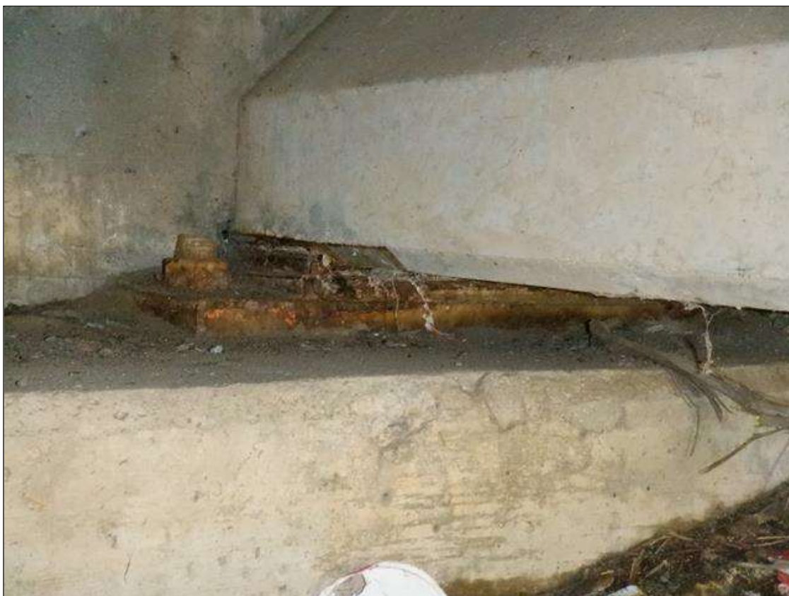
Span 1 Beam 1 - Near Bearing: RUST SCALE
