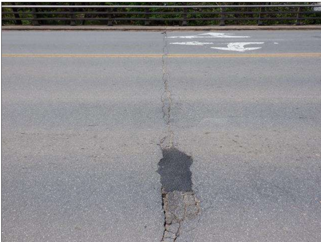
Span 3 Wearing Surface: 44 FEET X UP TO 2 INCHES TRANSVERSE CRACK AT BENT 2.
