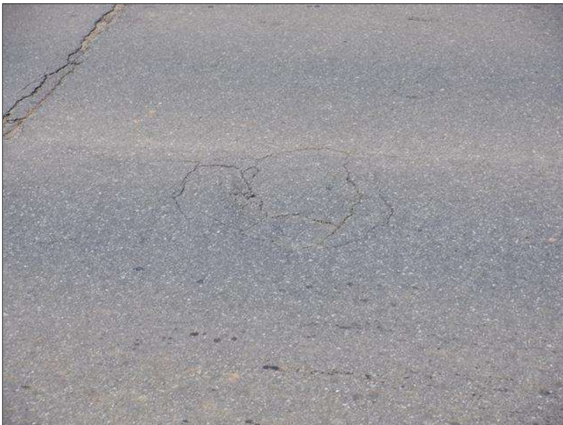
Span 2 Wearing Surface: 50 SQUARE FEET OF UP TO 1/16 INCHES MAP CRACKING AT RANDOM THROUGHOUT.
