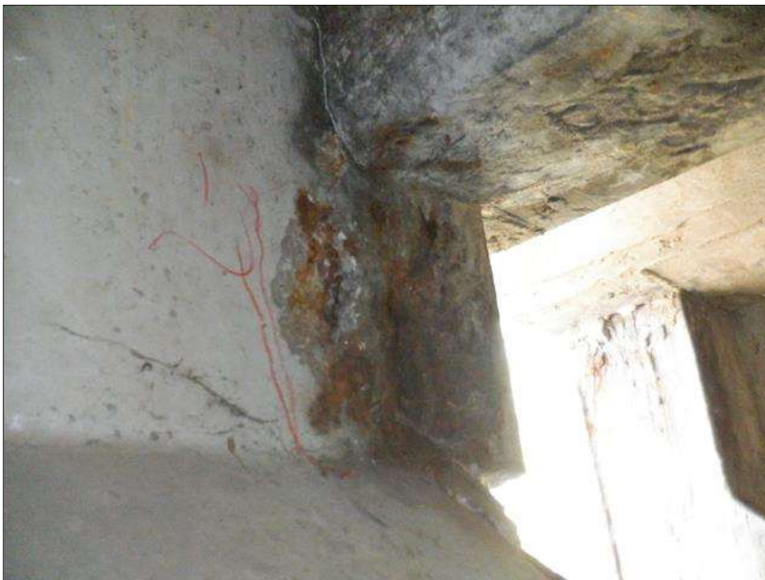
Span 2 Beam 8: 9 INCHES X UP TO 8 INCHES X 1 INCHES SPALL WITH EXPOSED REINFORCING ON WEST FACE OF WEB AT BENT 1.
