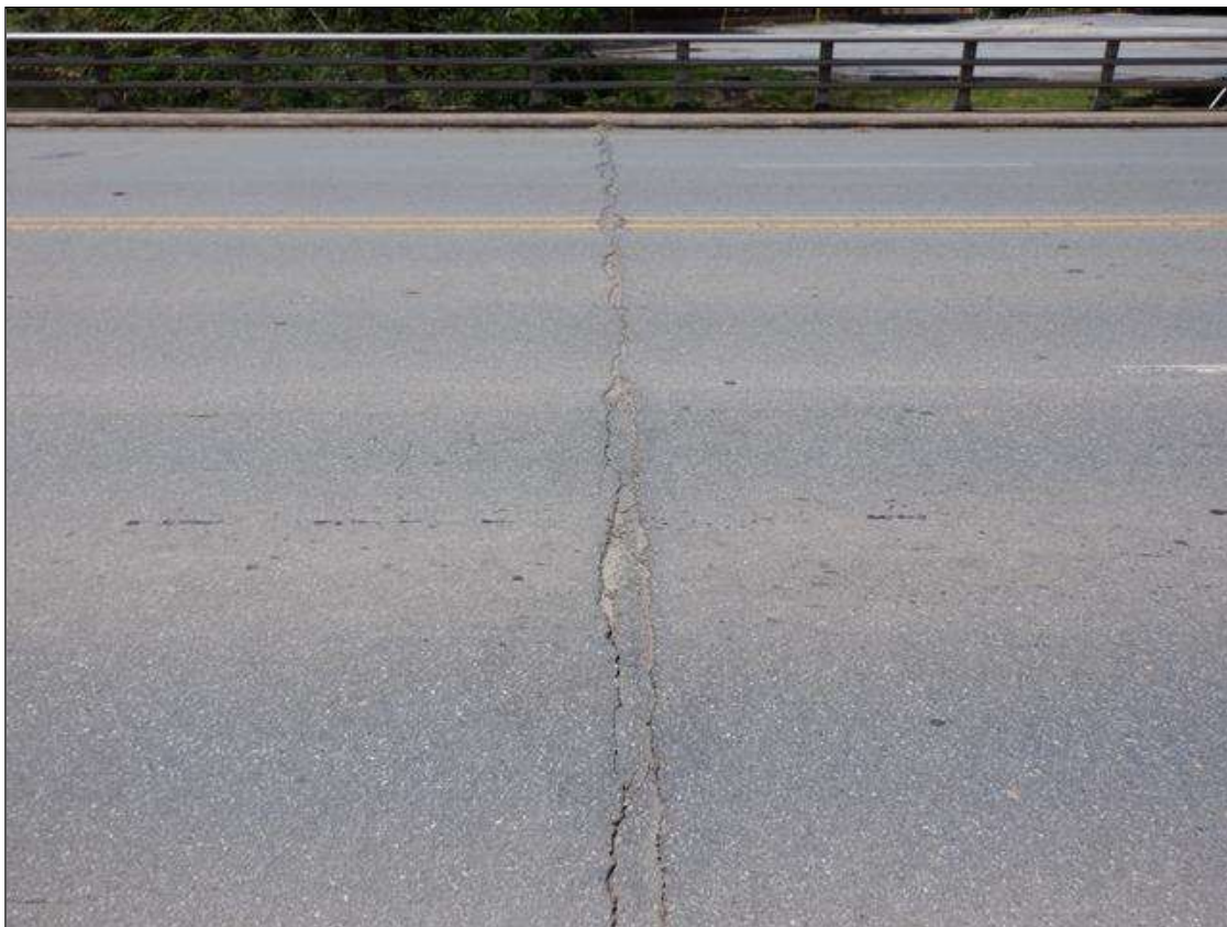
Span 4 Wearing Surface: 44 FEET X UP TO 3 INCHES TRANSVERSE CRACK AT BENT 3.
