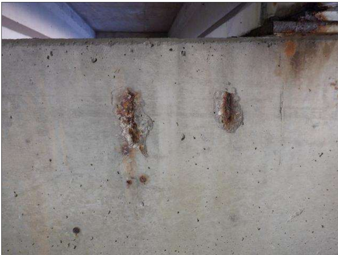
Bent 2 Cap 1: (2) UP TO 6 INCHES X 10 INCHES X 1 INCHES SPALLS WITH EXPOSED REINFORCING ON SOUTH FACE BETWEEN BEAMS 6 AND 7.
