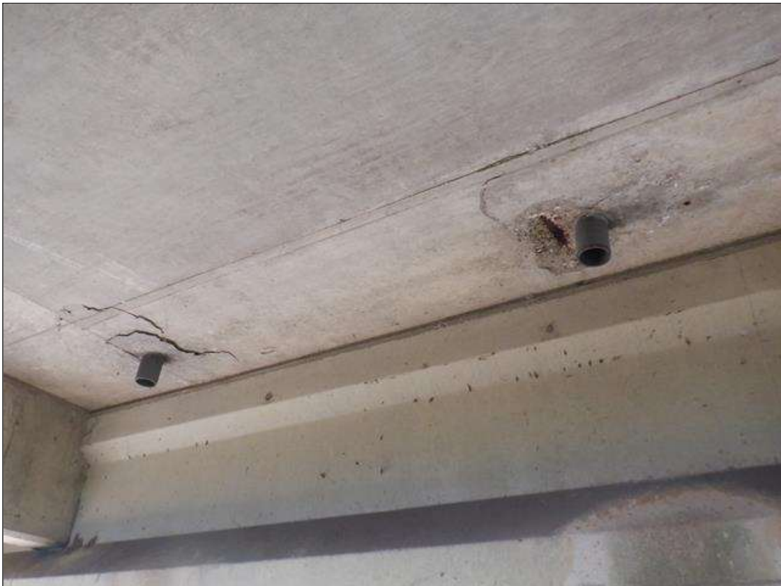
Span 2 Deck: 18 INCHES X UP TO 12 INCHES X 2 INCHES SPALL WITH EXPOSED REINFORCING ON DECK UNDERSIDE AROUND SECOND DRAIN BETWEEN BEAMS 1 AND 2 MEASURED FROM BENT 2.
