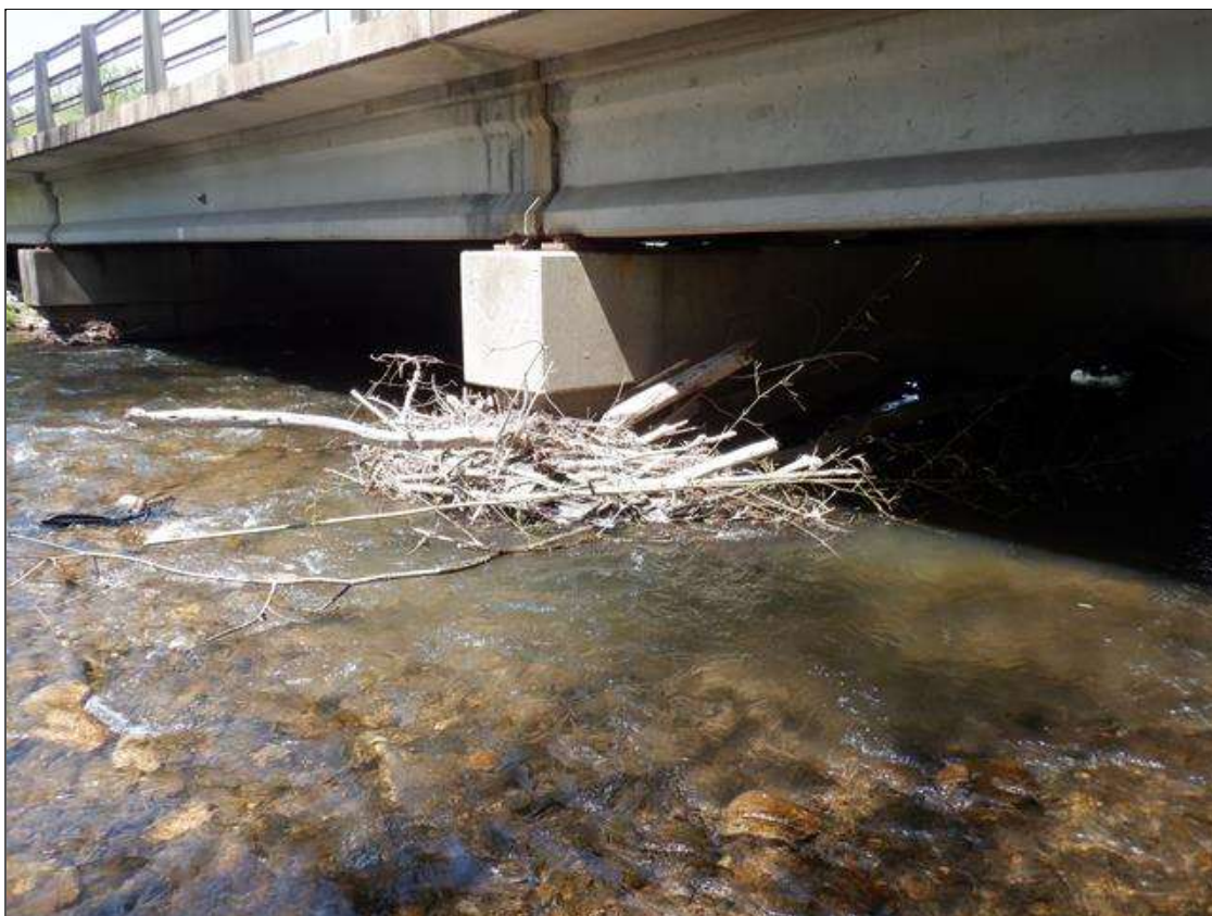
DRIFT: 45 FEET X UP TO 15 FEET X 4 FEET TIMBER DRIFT AND DEBRIS CAUGHT AT UPSTREAM END OF BENT 2.
