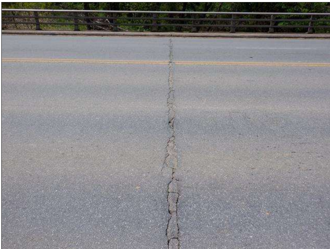
Span 2 Wearing Surface: 44 FEET X UP TO 3 INCHES TRANSVERSE CRACK AT BENT 1.
