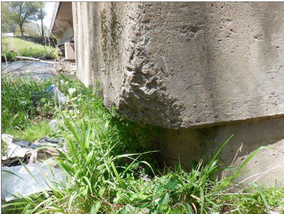
Bent 1 Cap 1: 10 INCHES X UP TO 10 INCHES X 10 INCHES SPALL ON SOUTHWEST CORNER OF SOUTH FACE.
