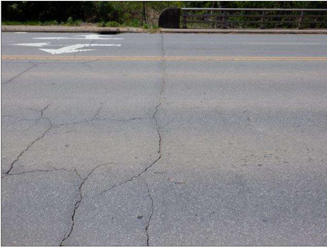
Span 1 Wearing Surface: 44 FEET X UP TO 1 INCHES TRANSVERSE CRACK AT END BENT 1.
