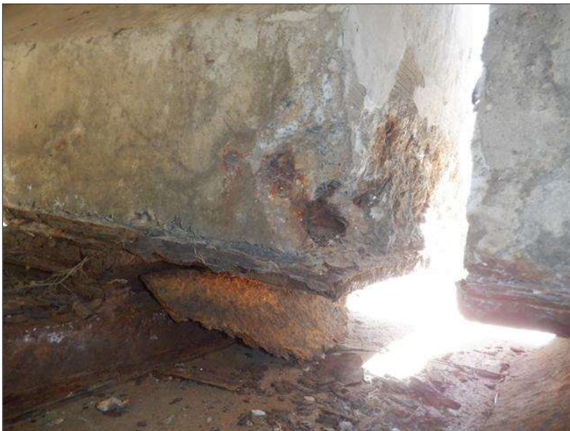
Span 2 Beam 1: (PAR) 3 INCHES X 5 INCHES X UP TO 18 INCHES SPALL WITH EXPOSED PRESTRESSED STRANDS ON THE NORTH FACE OF THE BOTTOM FLANGE AT BENT 2.
