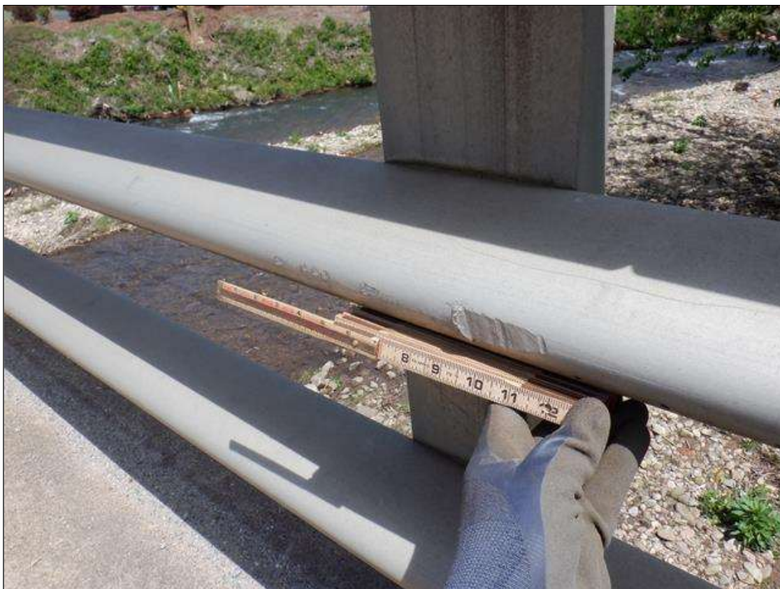
Span 2 Right Bridge Rail: 12 INCHES SCRAPE ON MID RAIL, 3 FEET FROM BENT 1.
