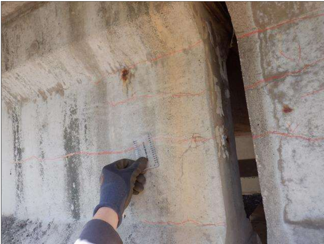
Span 3 Beam 1: (4) UP TO 3 FEET X 0.006 INCHES LONGITUDINAL CRACKS IN WEST FACE OF WEB EXTENDING FROM BENT 2.
