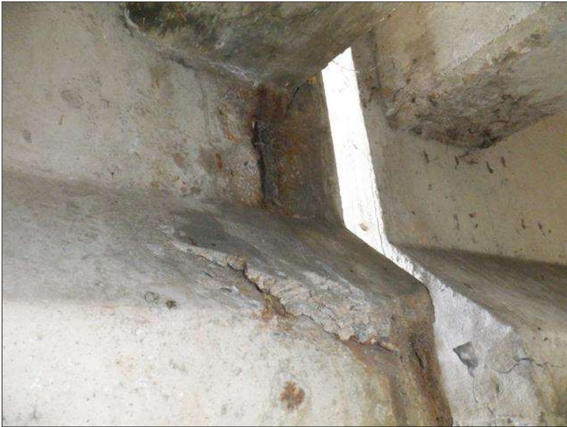
Span 4 Beam 8: (2) UP TO 14 INCHES X 16 INCHES X 1.5 INCHES SPALLS WITH EXPOSED REINFORCING ON WEST FACE OF BOTTOM FLANGE, CHAMFER, AND THE WEB AT BENT 3.
