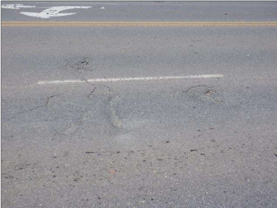
Span 3 Wearing Surface: (2) 2 FEET DIAMETER AREAS OF UP TO 1/2 INCHES ALLIGATOR CRACKING IN NORTHBOUND LANE.
