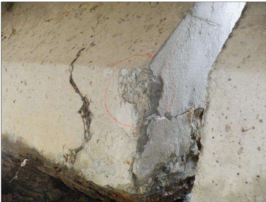
Span 3 Beam 1: 3 INCHES DIAMETER X 1/2 INCHES SPALL IN NORTHEAST CORNER OF BOTTOM FLANGE AT BENT 3
