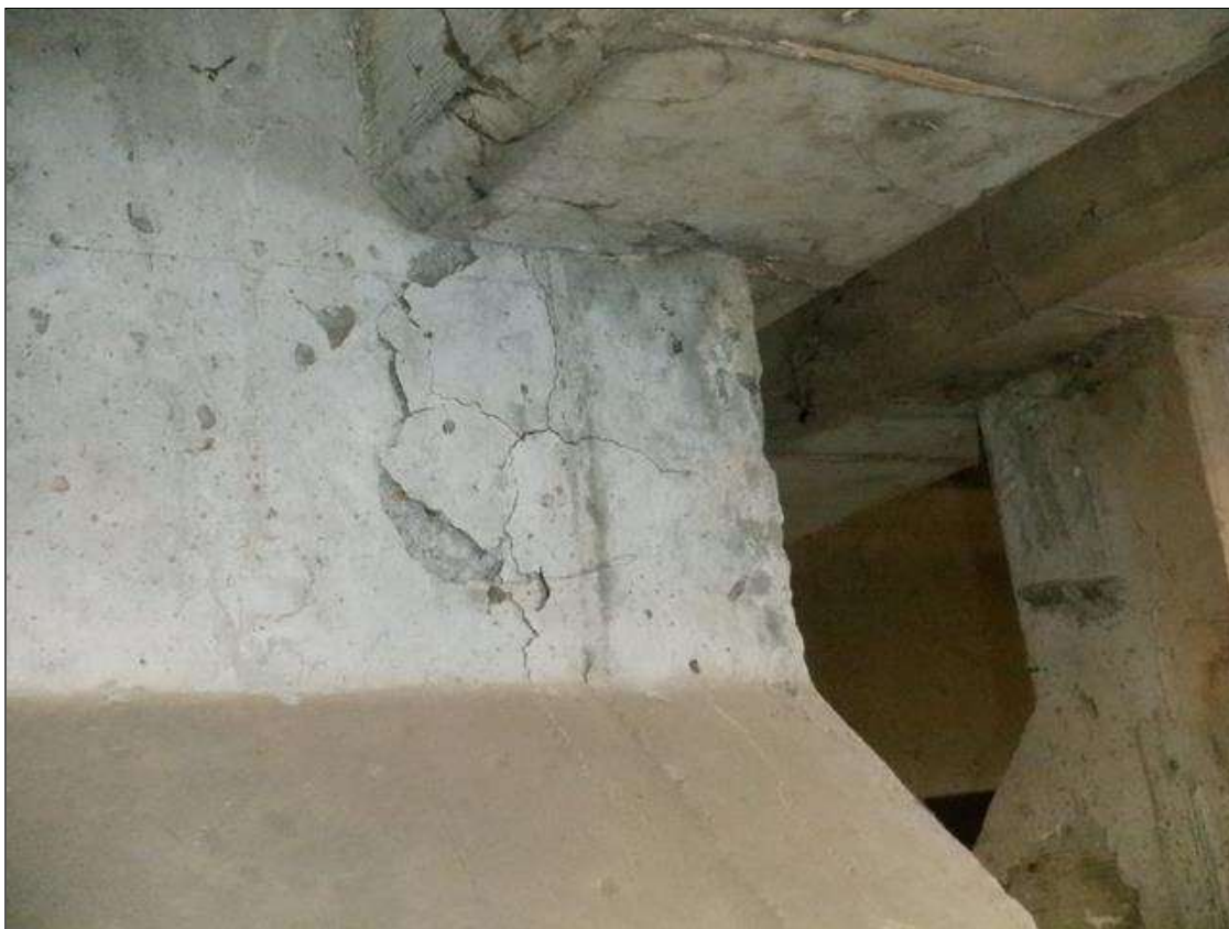
Span 1 Beam 5: 8 INCHES X UP TO 8 INCHES DELAMINATION WITH UP TO 0.006 INCHES MAP CRACKING ON EAST FACE AT BENT 1.
