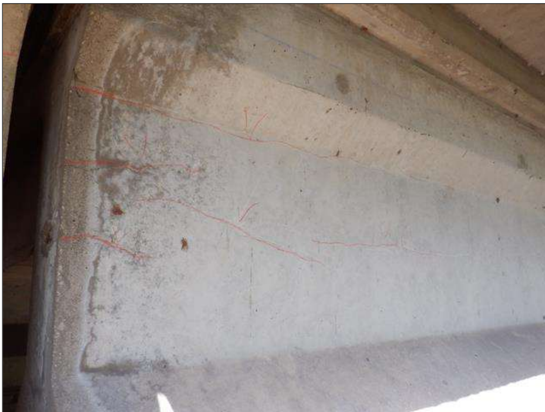
Span 2 Beam 1: (5) UP TO 4 FEET X 0.008 INCHES LONGITUDINAL CRACKS IN WEST WEB EXTENDING FROM BENT 2.
