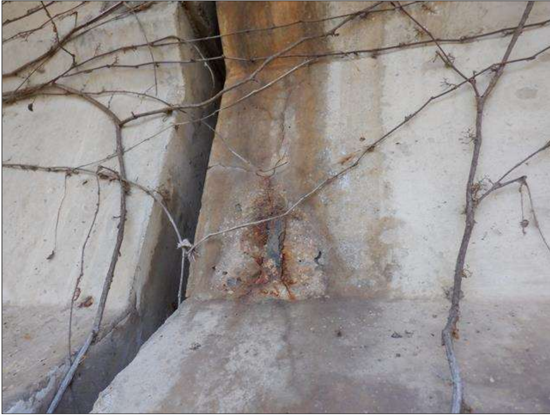
Span 4 Beam 8: 7 INCHES X 6 INCHES X UP TO 3/4 INCHES SPALL WITH EXPOSED REINFORCING WITH ADJACENT 8 INCHES X 10 INCHES AREA OF UP TO 0.008 INCHES MAP CRACKING ON EAST FACE OF WEB AT BENT 3.
