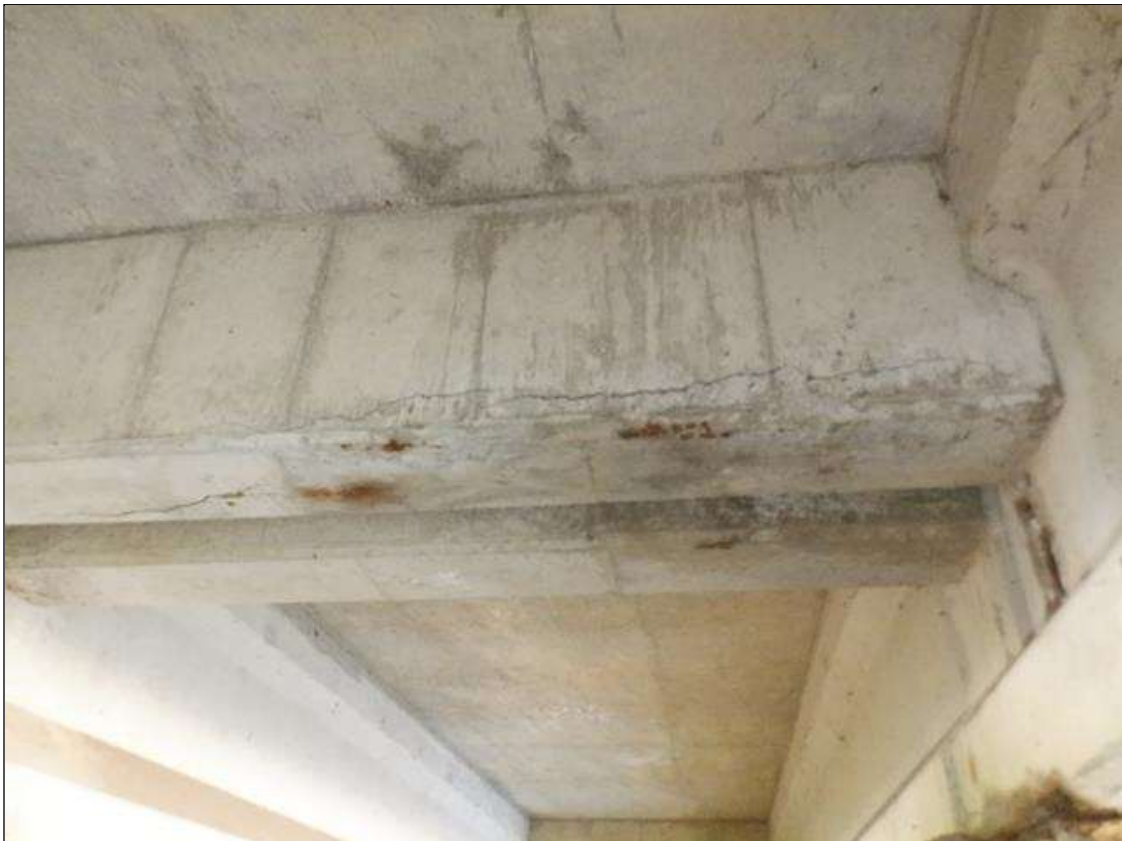
Span 2 Beam 7: 5 FEET X UP TO 10 INCHES CRACKED DELAMINATION WITH UP TO 1/4 INCHES CRACKING AND RUST STAINING ON BOTTOM FACE OF END DIAPHRAGM BETWEEN BEAMS 6 AND 7 AT BENT 2.
