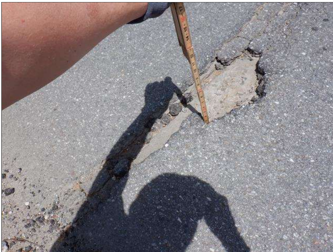
Span 3 Wearing Surface: 11 INCHES X UP TO 30 INCHES X FULL DEPTH POTHOLE IN SOUTHBOUND LANE AT BENT 2, 18 INCHES FROM WEST CURB.
