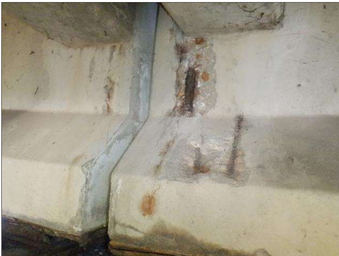
Span 2 Beam 7: (PAR) (5) UP TO 13 INCHES X 0.02 INCHES VERTICAL CRACKS WITH RUST STAINING ON WEST FACE OF THE WEB, CHAMFER, AND BOTTOM FLANGE AT BENT 2.
