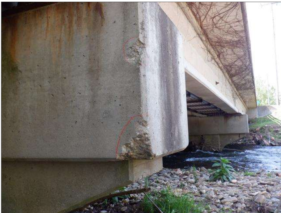
Bent 2 Cap 1: (2) UP TO 6 INCHES X 6 INCHES X 6 INCHES SPALLS ON SOUTHEAST CORNER AT EAST END.
