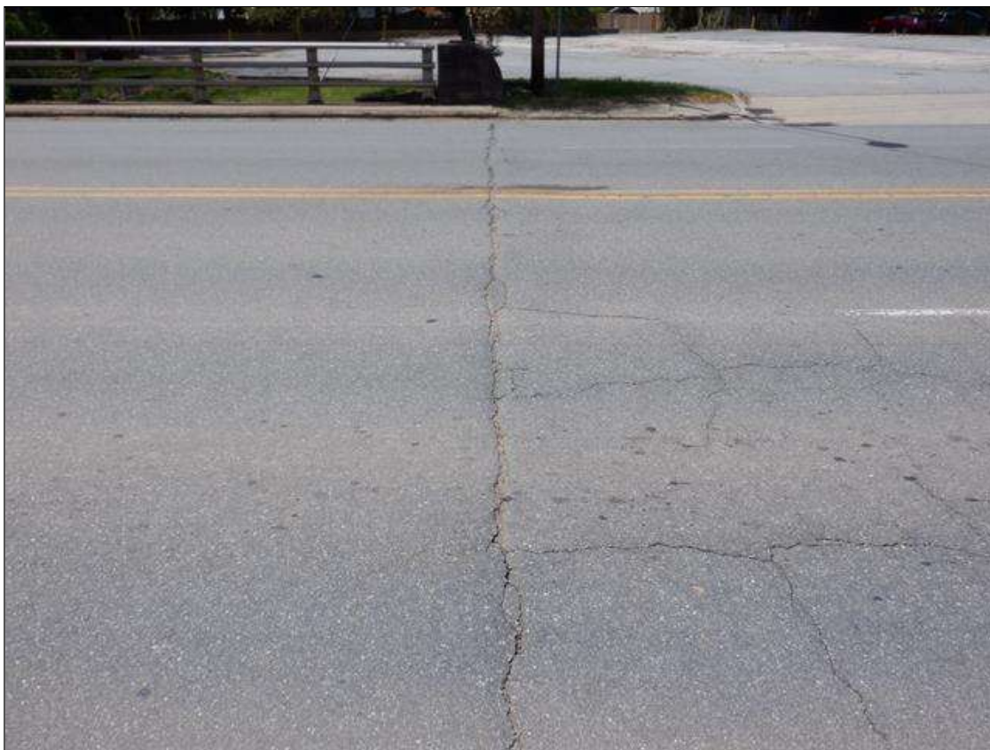
Span 4 Wearing Surface: 44 FEET X UP TO 1 INCHES TRANSVERSE CRACK AT END BENT 2.
