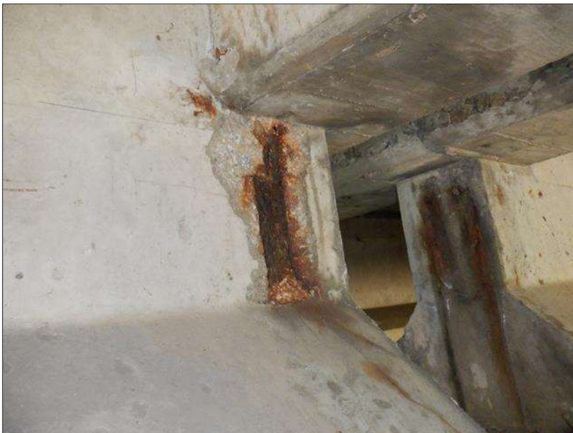
Span 2 Beam 3: 4 INCHES X UP TO 6 INCHES X 1 INCHES SPALL WITH EXPOSED REINFORCING ON WEST FACE AT BENT 1.
