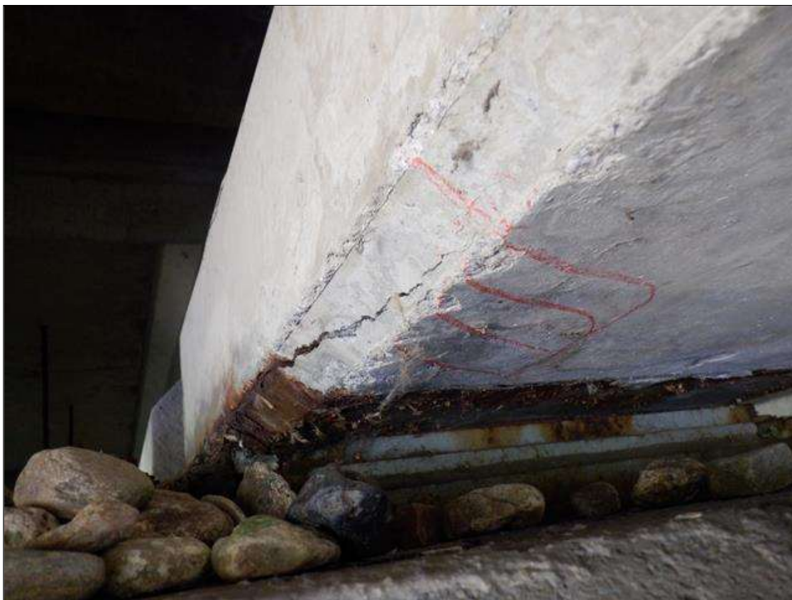
Span 2 Beam 7: (PAR) 8 INCHES X UP TO 0.1 INCHES LONGITUDINAL CRACK WITH ADJACENT 4 INCHES X UP TO 4 INCHES DELAMINATION ON THE EAST FACE OF THE BOTTOM FLANGE AND THE BOTTOM FACE AT BENT 1.
