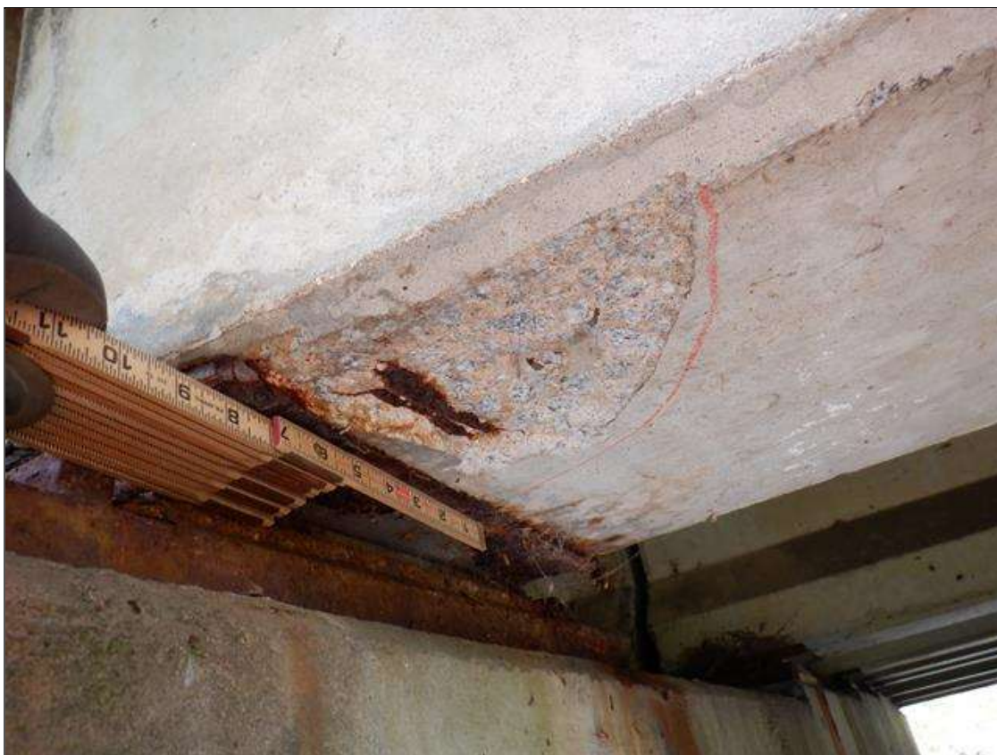
Span 3 Beam 1: 8 INCHES DIAMETER X UP TO 1/2 INCHES SPALL IN UNDERSIDE OF BOTTOM FLANGE, 15 INCHES FROM BENT 3.
