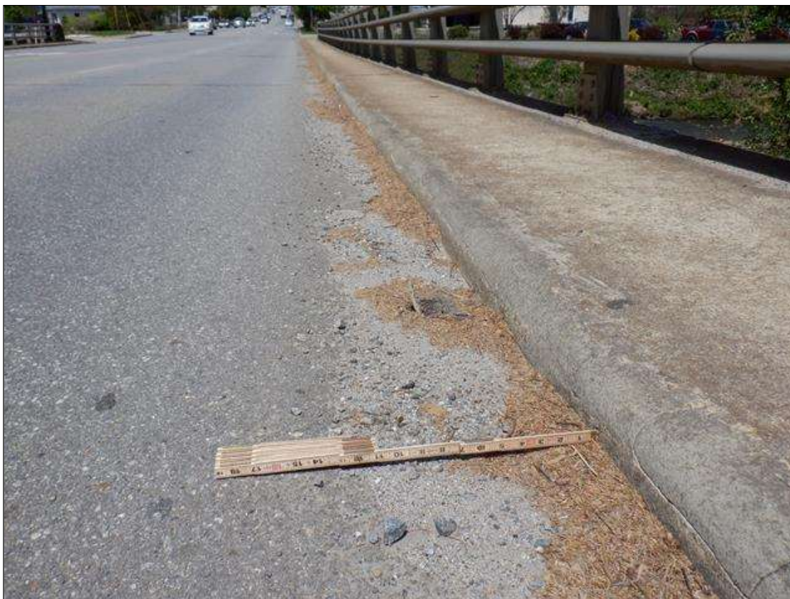
DECK DEBRIS: FULL LENGTH X 14 INCHES X UP TO 2 INCHES SEDIMENT AND DEBRIS IN EAST GUTTER (WEST GUTTERS SIMILAR)
