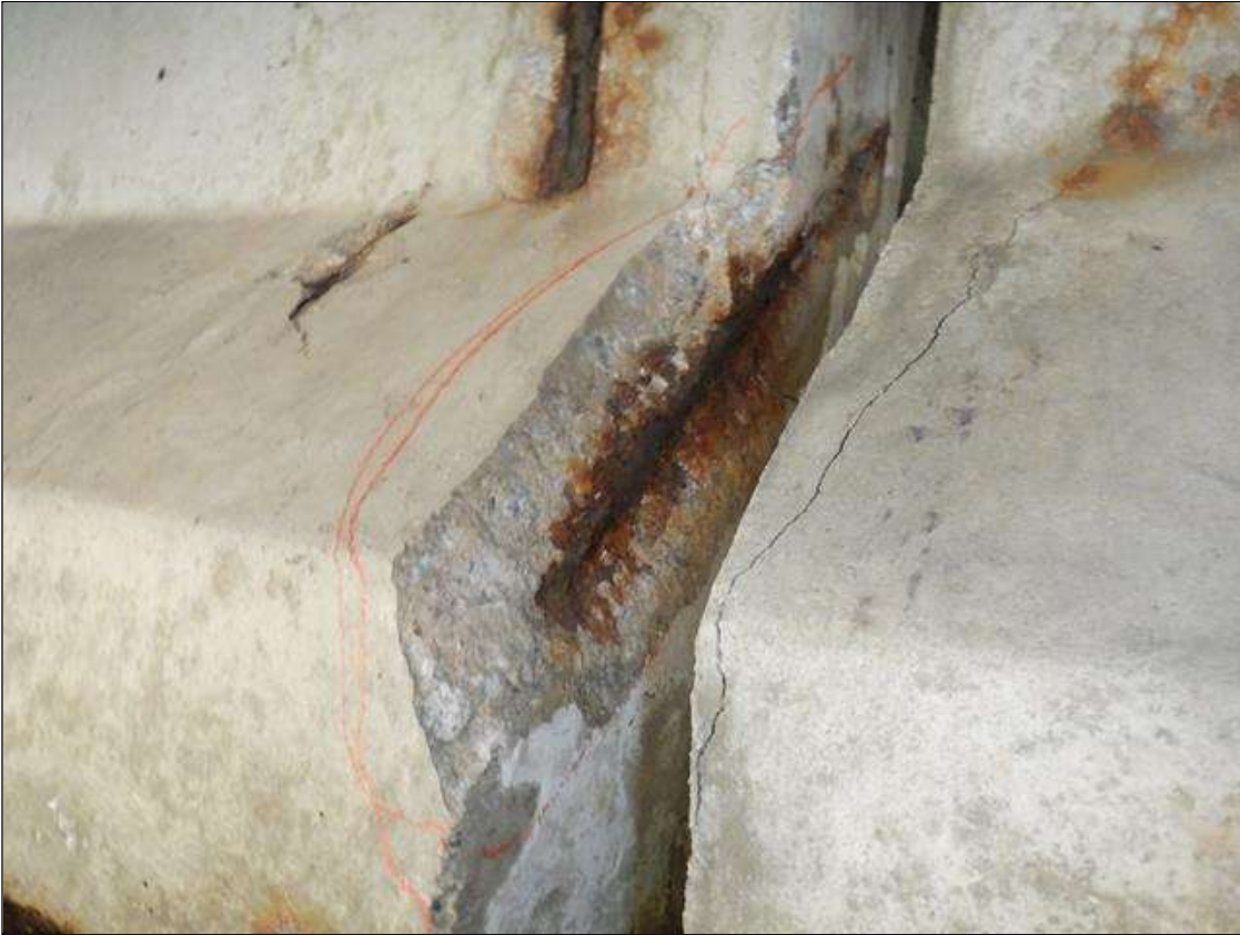
Span 2 Beam 6: 2 INCHES X UP TO 14 INCHES X 1.5 INCHES SPALL WITH EXPOSED REINFORCING IN NORTH FACE OF BOTTOM FLANGE AND CHAMFER AT BENT 2.
