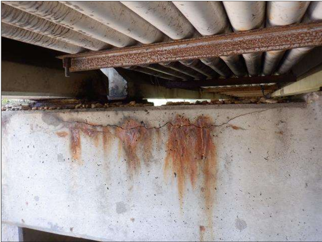
Bent 1 Cap 1: 43 INCHES X UP TO 1/8 INCHES LONGITUDINAL CRACK WITH RUST STAINING ON NORTH FACE BETWEEN BEAMS 7 AND 8.
