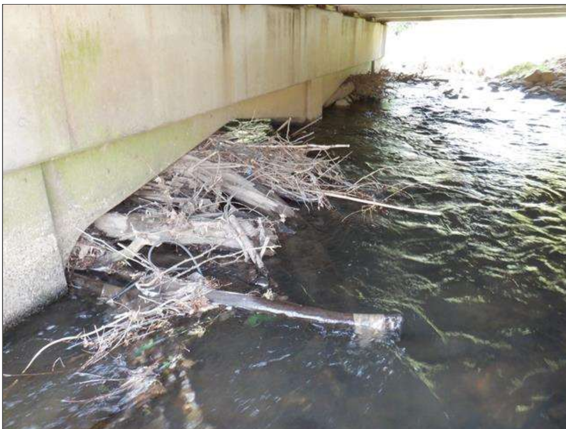
DRIFT: (3) UP TO 12 FEET X 10 FEET X 3 FEETS AREAS OF LOGS AND DEBRIS CAUGHT ALONG AND UNDER BENT 3.
