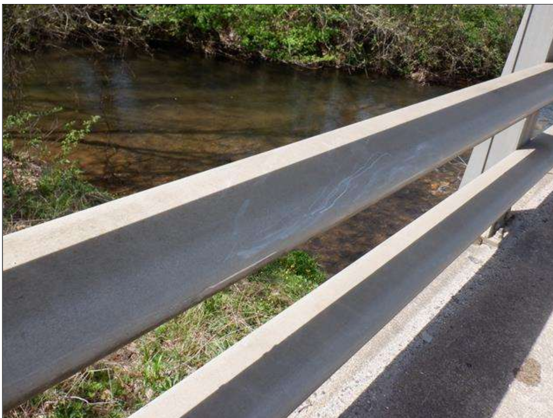
Span 2 Left Bridge Rail: (3) UP TO 2 FEET SCRAPES ON THE MID RAIL, 6 FEET FROM BENT 1.
