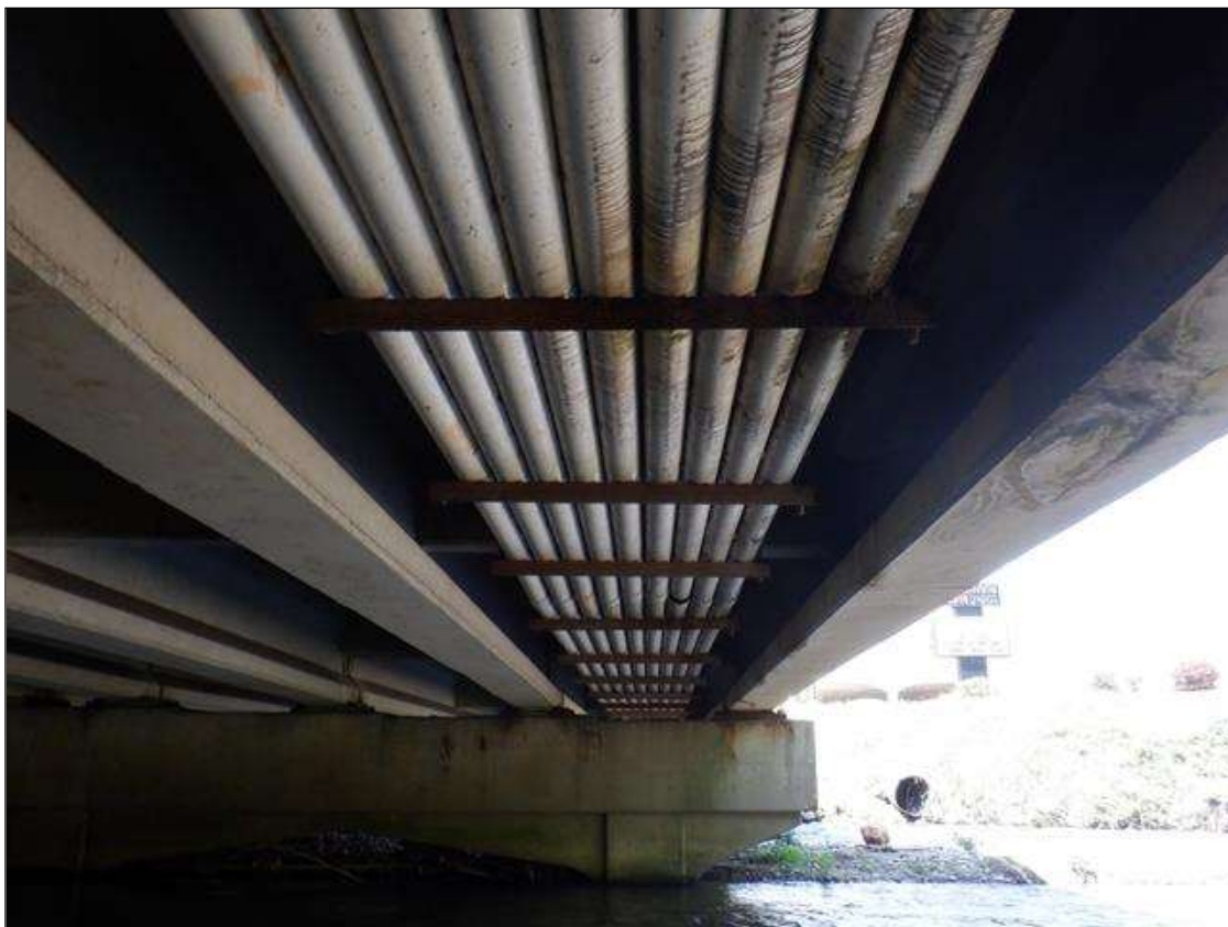
UTILITY: (9) 4 INCHES DIAMETER PVC CONDUITS ATTACHED TO UNDERSIDE OF BAY 7
