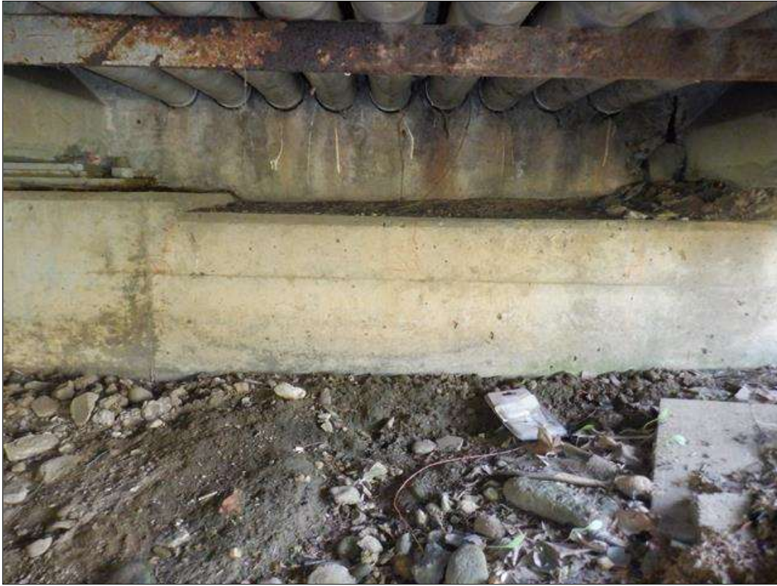
End Bent 2 Cap 1: (3) UP TO 10 INCHES X 1/64 INCHES VERTICAL CRACKS ON SOUTH FACE BETWEEN BEAMS 7 AND 8.
