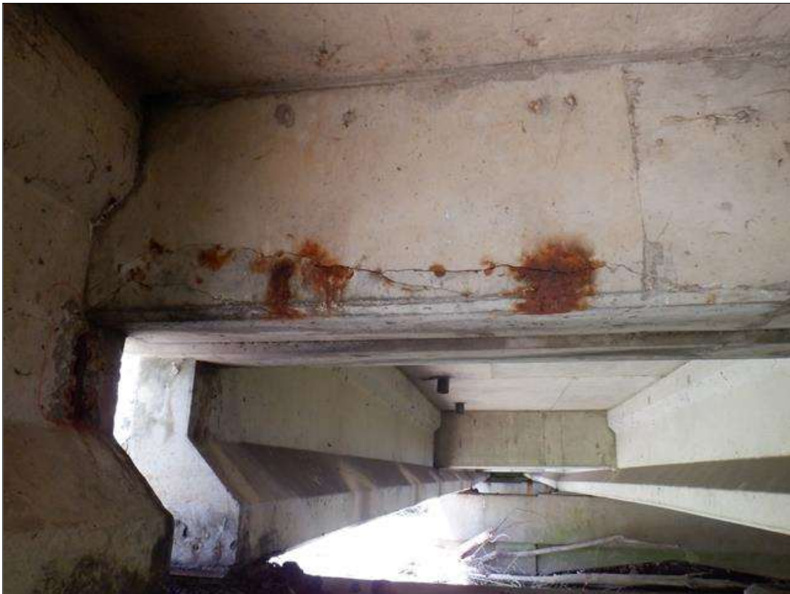
Span 1 Beam 1: 4 FEET X UP TO 8 INCHES CRACKED DELAMINATION WITH UP TO 0.063 INCHES CRACKING AND RUST STAINING ON SOUTH FACE OF END DIAPHRAGM BETWEEN BEAMS 1 AND 2 AT BENT 1.
