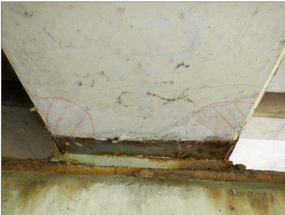
Span 4 Beam 2: (2) UP TO 3 INCHES DIAMETER DELAMINATIONS ON BOTTOM FACE, 2 FEET FROM BENT 3.
