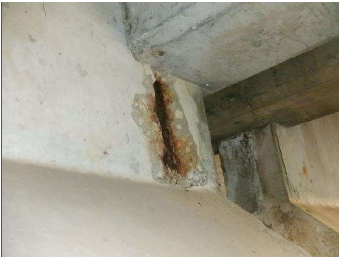
Span 1 Beam 7: 6 INCHES X UP TO 8 INCHES X 1 INCHES SPALL WITH EXPOSED REINFORCING ON EAST FACE AT BENT 1.
