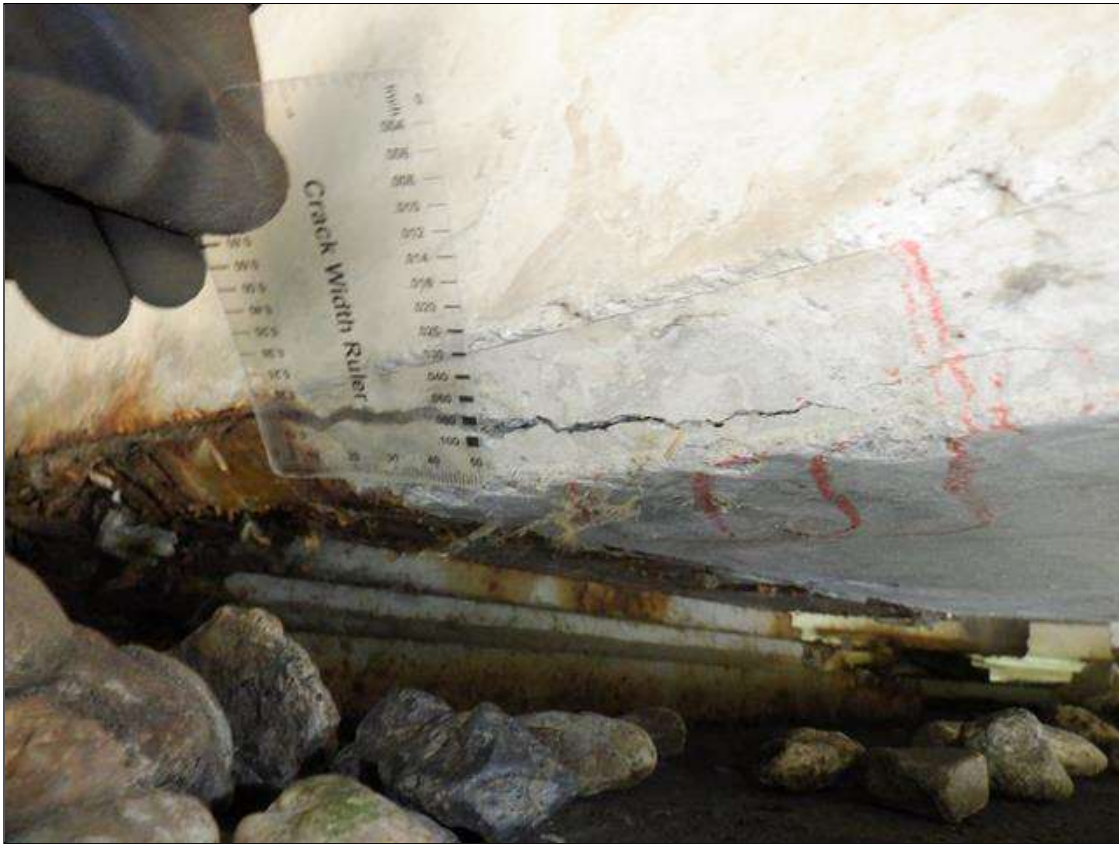
Span 2 Beam 7: (PAR) 8 INCHES X UP TO 0.1 INCHES LONGITUDINAL CRACK WITH ADJACENT 4 INCHES X UP TO 4 INCHES DELAMINATION ON THE EAST FACE OF THE BOTTOM FLANGE AND THE BOTTOM FACE AT BENT 1.
