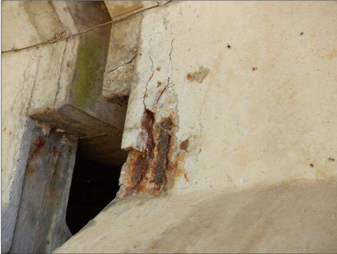
Span 2 Beam 8: 6 INCHES X 7 INCHES X UP TO 1 INCHES SPALL WITH EXPOSED REINFORCING WITH ADJACENT 9 INCHES X 14 INCHES DELAMINATION AND UP TO 0.008 INCHES VERTICAL CRACKS ON EAST FACE OF WEB AT BENT 1.
