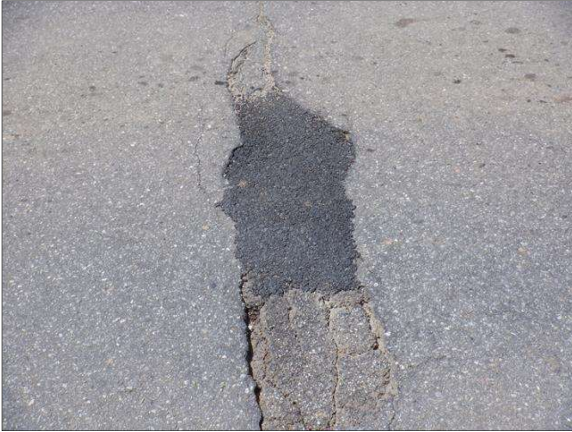
Span 3 Wearing Surface: 1 FEET X 3 FEET ASPHALT PATCH AT BENT 2, 5 FEET FROM EAST CURB
