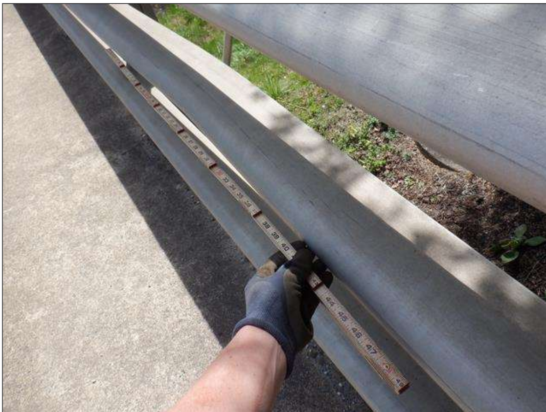
Span 4 Left Bridge Rail: 4 FEET X UP TO 1 INCHES DISTORTION OF THE MID RAIL, 5 FEET FROM END BENT 2.
