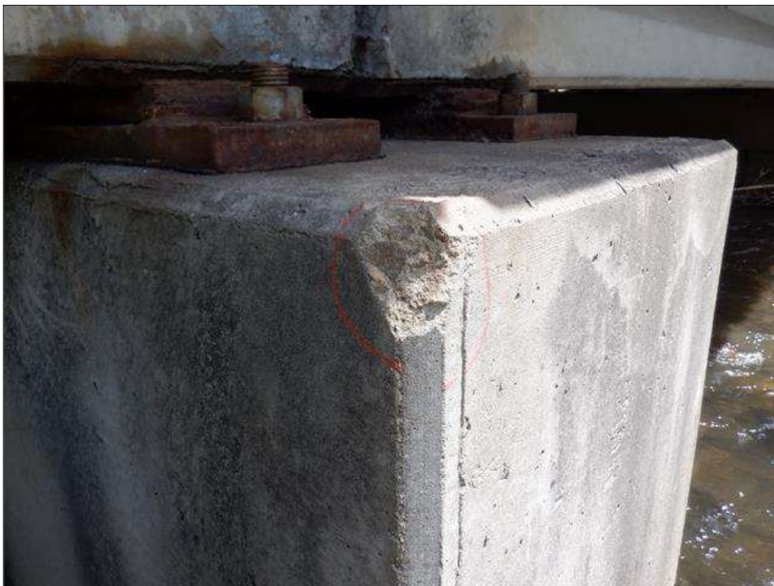
Bent 3 Cap 1: 3 INCHES DIAMETER X 1/2 INCHES SPALL IN TOP OF NORTHWEST CORNER.
