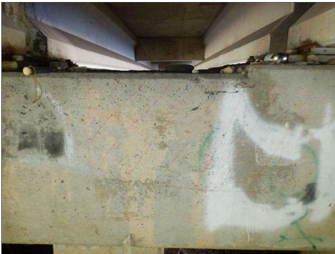
Bent 1 Cap 1: 3 FEET X UP TO 2 FEET DELAMINATION WITH UP TO 1/32 INCHES LONGITUDINAL CRACKS ON SOUTH FACE BELOW BAY 3.
