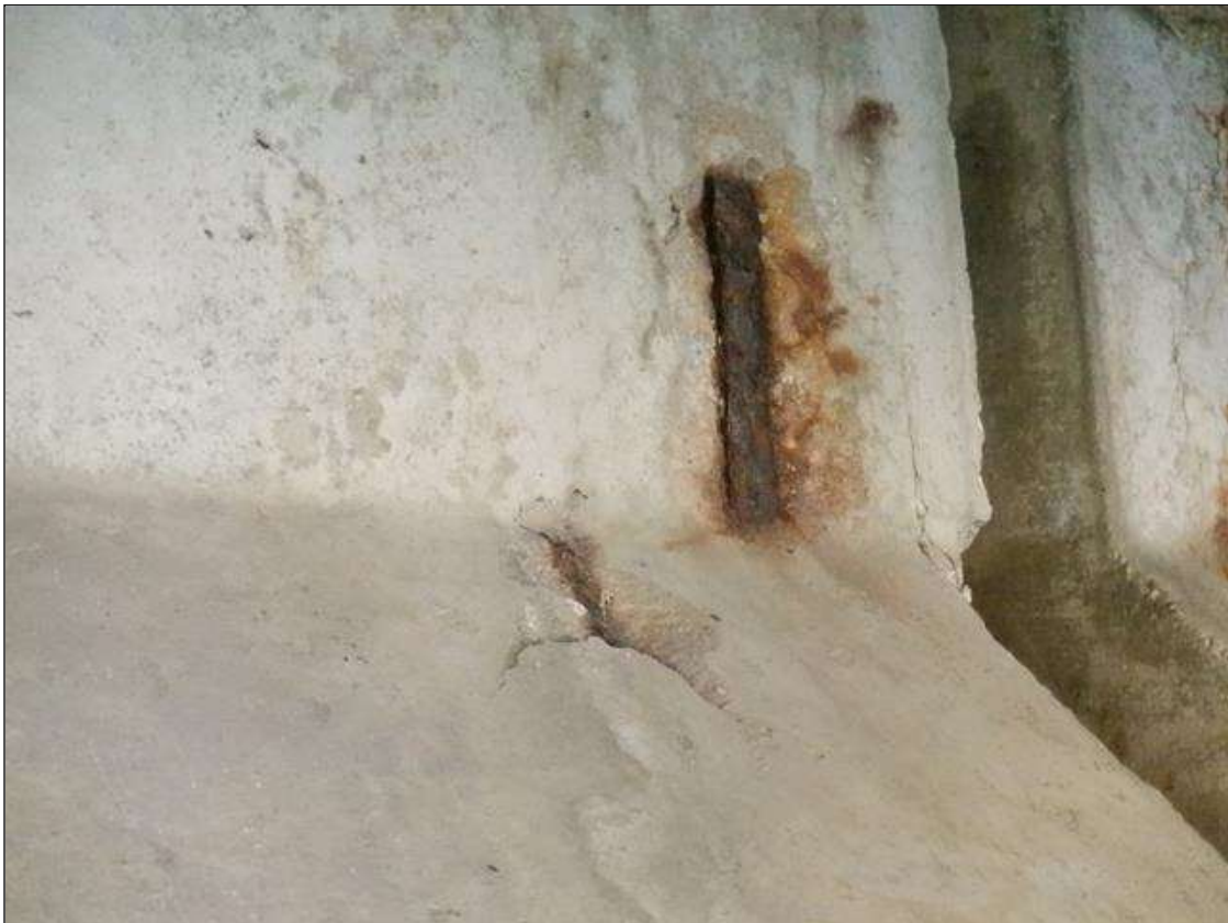
Span 2 Beam 6: (4) UP TO 6 INCHES X 4 INCHES X 1 INCHES SPALLS WITH EXPOSED REINFORCING ON EAST AND WEST FACES AT BENT 2.
