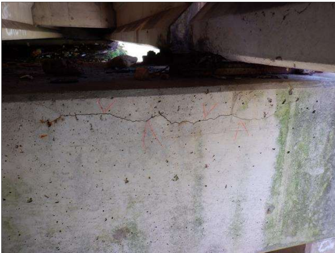
Bent 1 Cap 1: 3 FEET X UP TO 1/16 INCHES LONGITUDINAL CRACK ON NORTH FACE BETWEEN BEAMS 1 AND 2.
