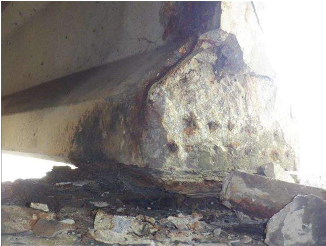
Span 2 Beam 8: (PAR) 7 INCHES X UP TO 1 FEET X 16 INCHES SPALL WITH EXPOSED REBAR AND PRESTRESSING STRANDS ON THE WEST AND SOUTH FACES OF BOTTOM FLANGE AND CHAMFER AT BENT 1.
