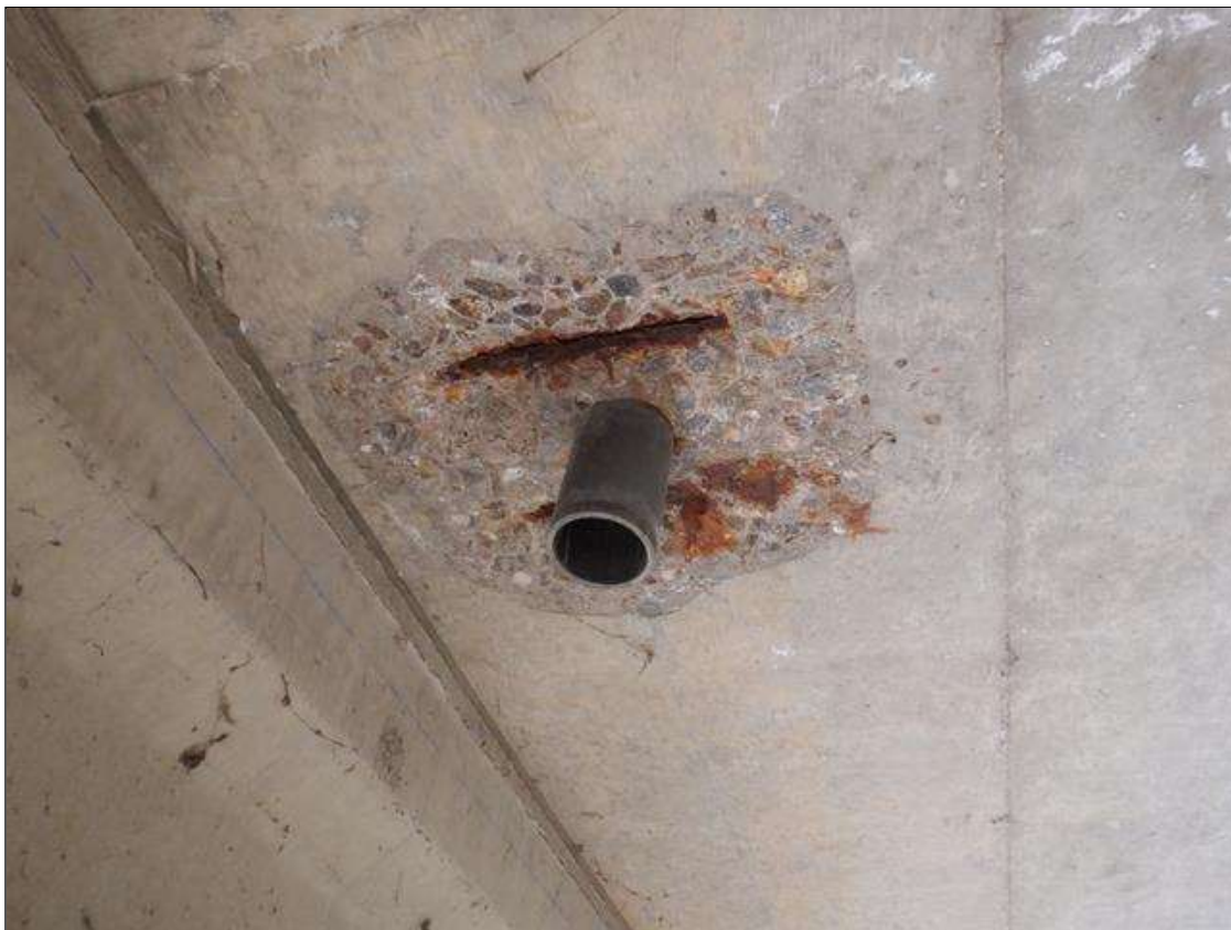
Span 3 Deck: 2 FEET X UP TO 2 FEET X 1 INCHES SPALL WITH EXPOSED REINFORCING ON DECK UNDERSIDE AROUND FIRST DRAIN BETWEEN BEAMS 1 AND 2 MEASURED FROM BENT 2.
