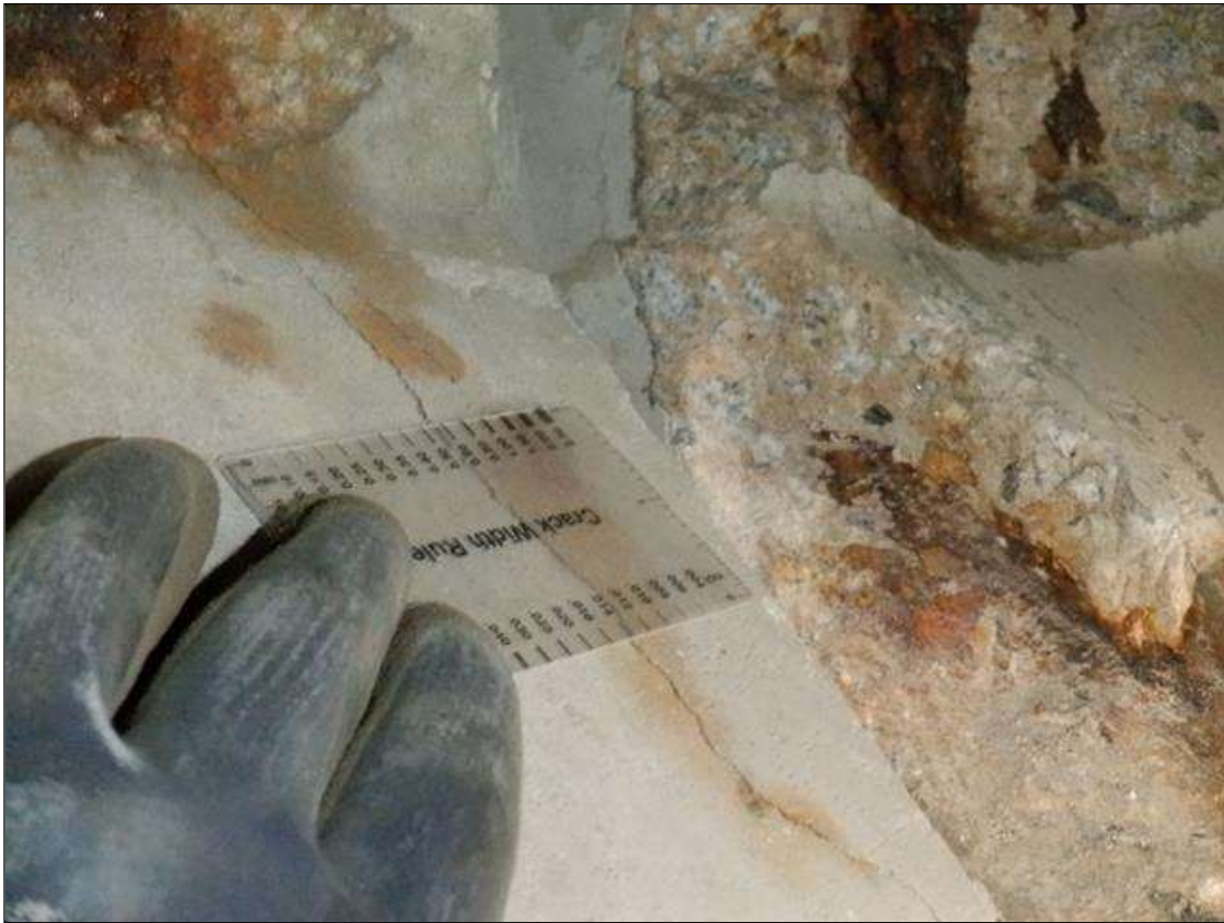
Span 2 Beam 7: (PAR) (2) UP TO 9 INCHES X 0.014 DIAGONAL CRACKS WITH RUST STAINING ON THE EAST FACE OF THE CHAMFER AND BOTTOM FLANGE AT BENT 2.
