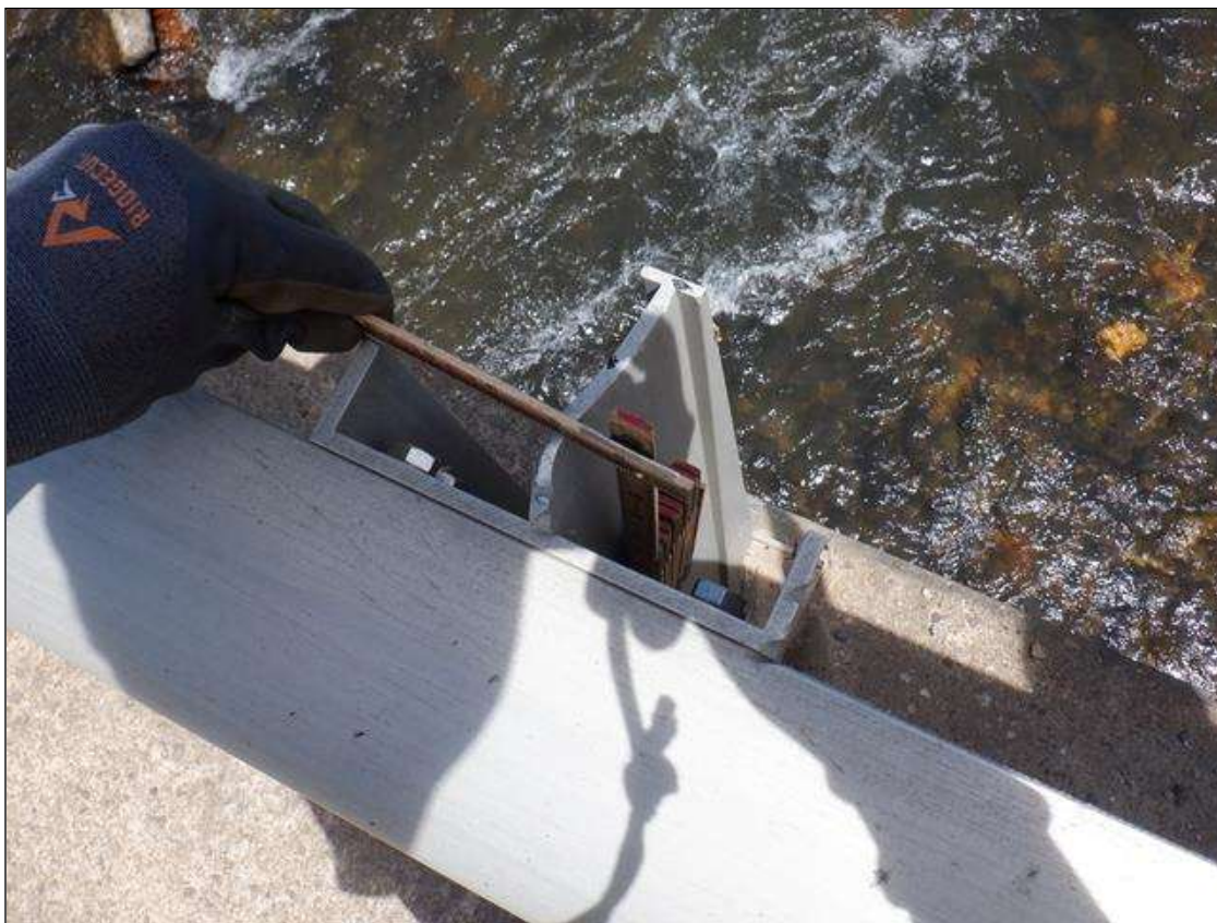
Span 3 Right Bridge Rail: UP TO 1/2 INCHES DISTORTION ON TOP OF SECOND RAIL POST MEASURED FROM BENT 3.
