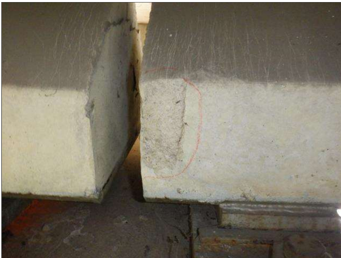
Span 3 Beam 2: 3 INCHES X 5 INCHES X 1/2 INCHES SPALL ON EAST FACE OF BOTTOM FLANGE AT BENT 2.
