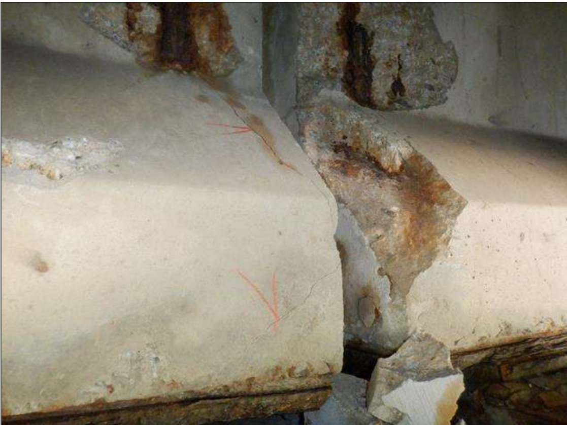
Span 2 Beam 7: (PAR) (2) UP TO 9 INCHES X 0.014 DIAGONAL CRACKS WITH RUST STAINING ON THE EAST FACE OF THE CHAMFER AND BOTTOM FLANGE AT BENT 2.
