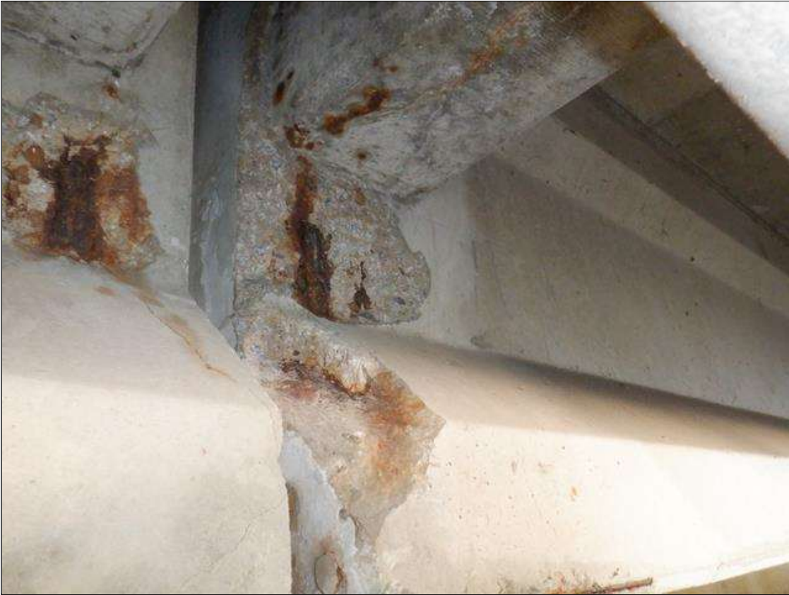
Span 3 Beam 7: (PAR) 12 INCHES X UP TO 20 INCHES X 4 INCHES SPALL WITH EXPOSED REINFORCING AND PRESTRESSED STRANDS ON THE EAST FACE AT BENT 2.
