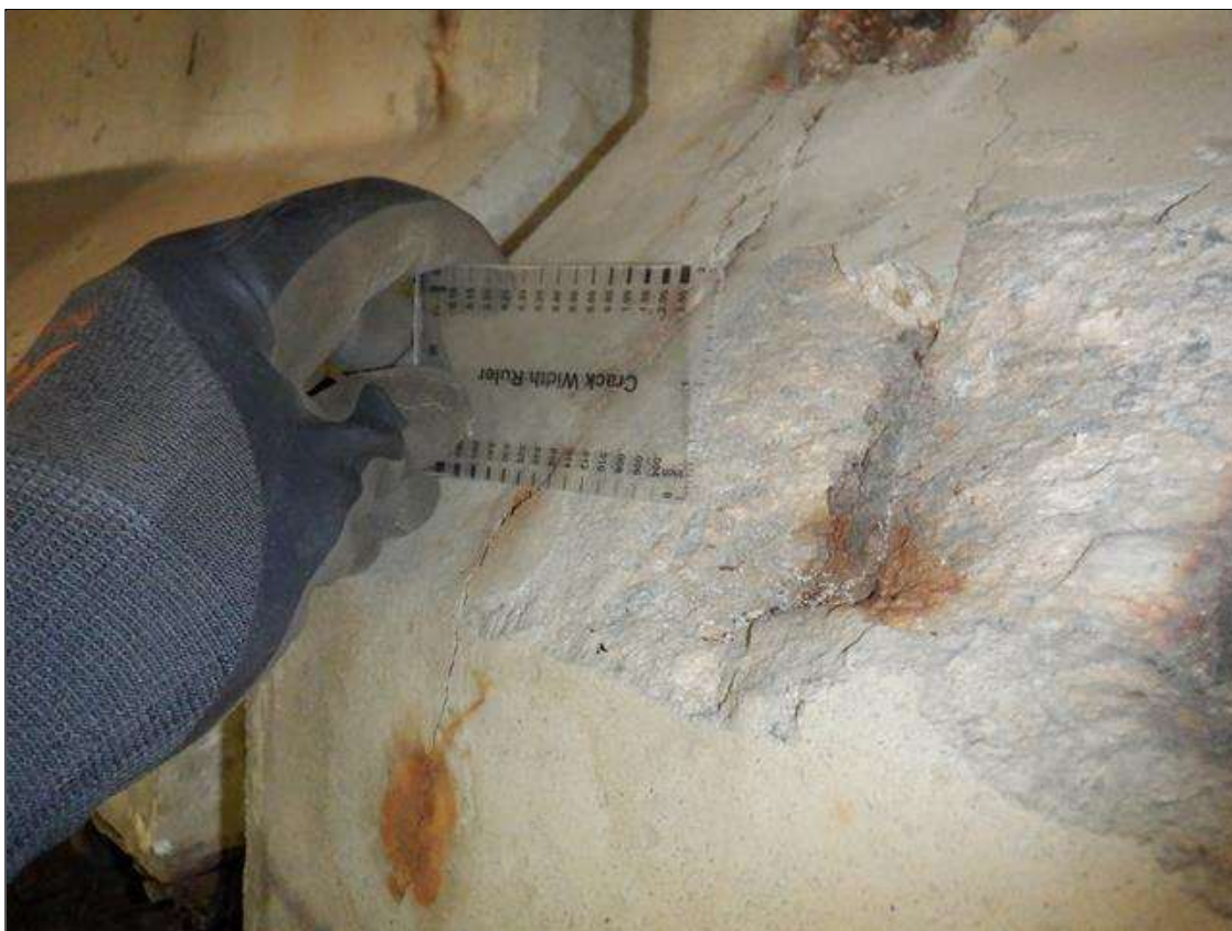
Span 2 Beam 7: (PAR) (5) UP TO 13 INCHES X 0.02 INCHES VERTICAL CRACKS WITH RUST STAINING ON WEST FACE OF THE WEB, CHAMFER, AND BOTTOM FLANGE AT BENT 2.
