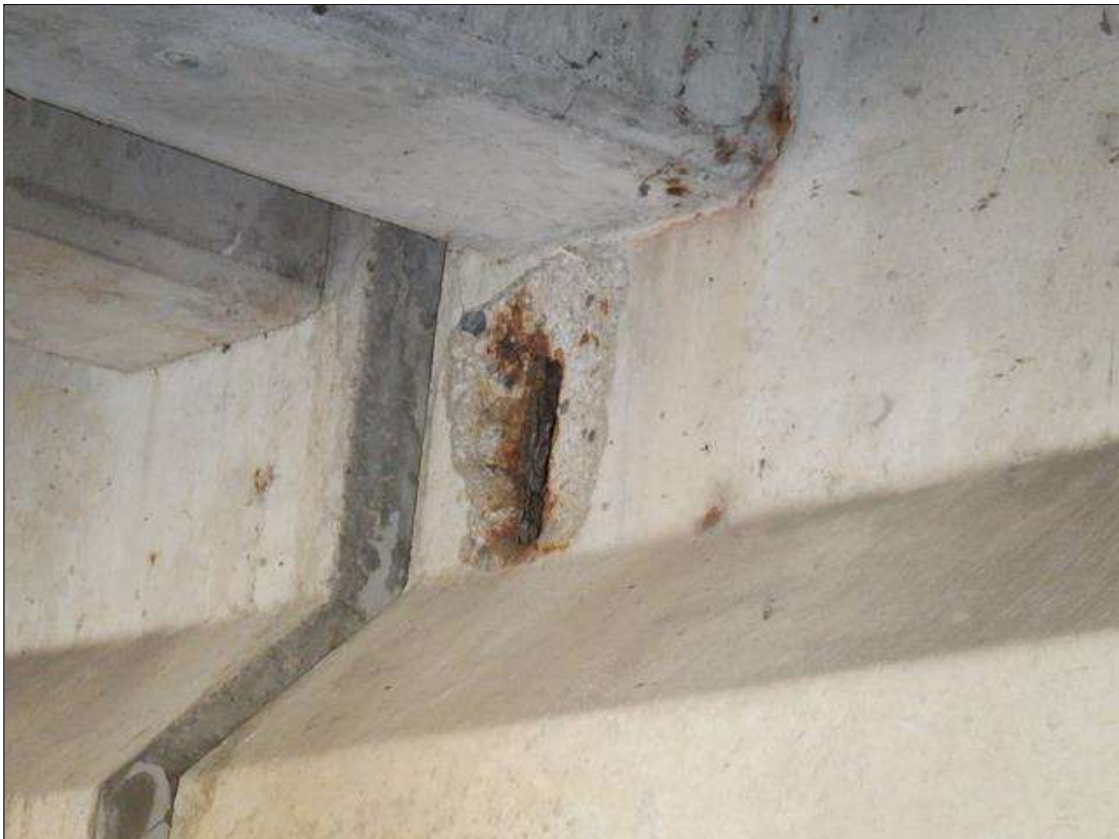
Span 4 Beam 6: 6 INCHES X UP TO 8 INCHES X 1 INCHES SPALL WITH EXPOSED REINFORCING ON EAST FACE AT BENT 3.
