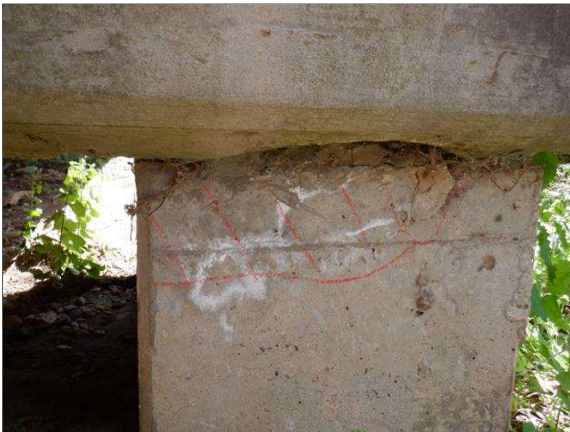
Bent 1 Pile 1: 6 INCHES X UP TO 18 INCHES DELAMINATION ON NORTH FACE AT BOTTOM OF CAP.
