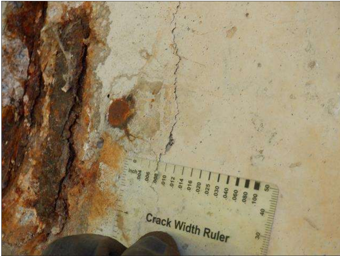
Span 2 Beam 8: 6 INCHES X 7 INCHES X UP TO 1 INCHES SPALL WITH EXPOSED REINFORCING WITH ADJACENT 9 INCHES X 14 INCHES DELAMINATION AND UP TO 0.008 INCHES VERTICAL CRACKS ON EAST FACE OF WEB AT BENT 1.
