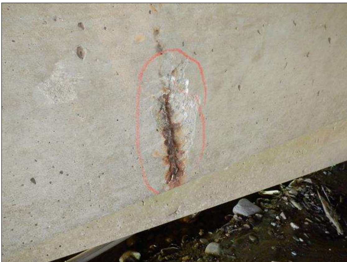
Bent 2 Cap 1: 3 INCHES X UP TO 6 INCHES X 1/2 INCHES SPALL WITH EXPOSED REINFORCING ON NORTH FACE BENEATH BEAM 6.
