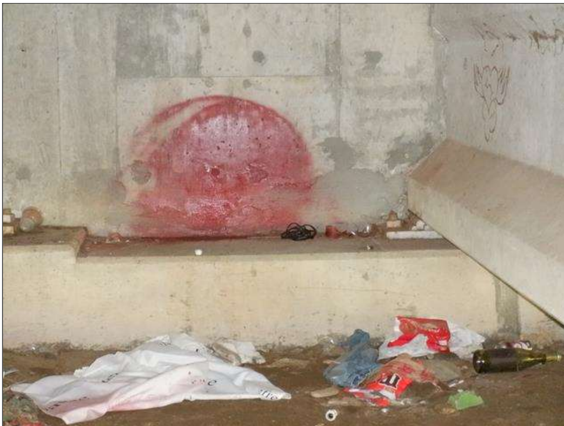
End Bent 1 Abutment: 5 FEET X 1 FEET PATCHED AREA ON NORTH FACE BETWEEN BEAMS 3 AND 4.
