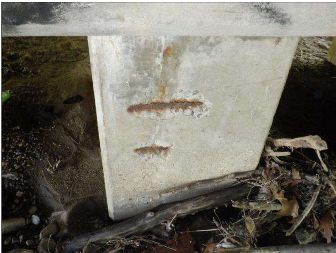
Bent 1 Pile 4: (2) UP TO 4 INCHES X 12 INCHES X 1 INCHES SPALLS WITH EXPOSED REINFORCING ON NORTH FACE, 1 FEET FROM BOTTOM OF CAP.
