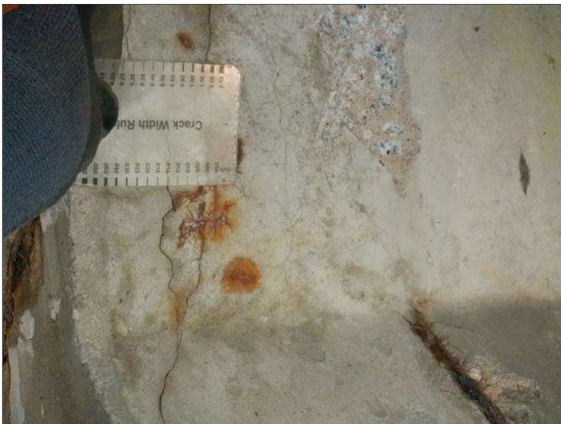
Span 2 Beam 6: (PAR) 5 INCHES X UP TO 11 INCHES AREA OF UP TO 0.014 INCHES MAP CRACKING WITH RUST STAINING ON THE WEST FACE OF THE WEB AND CHAMFER AT BENT 2.
