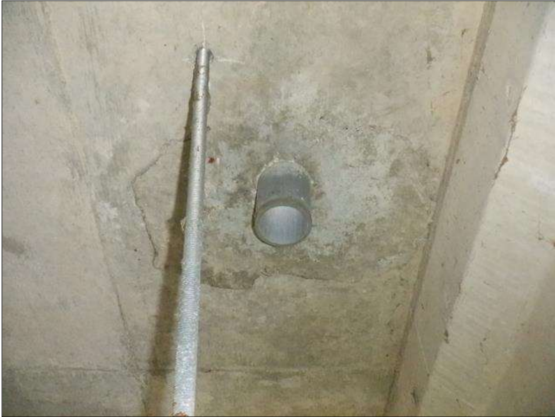
Span 2 Deck: 10 SQUARE FEET OF DELAMINATIONS ON DECK UNDERSIDE AT RANDOM THROUGHOUT DRAIN LOCATIONS BETWEEN BEAMS 7 AND 8.
