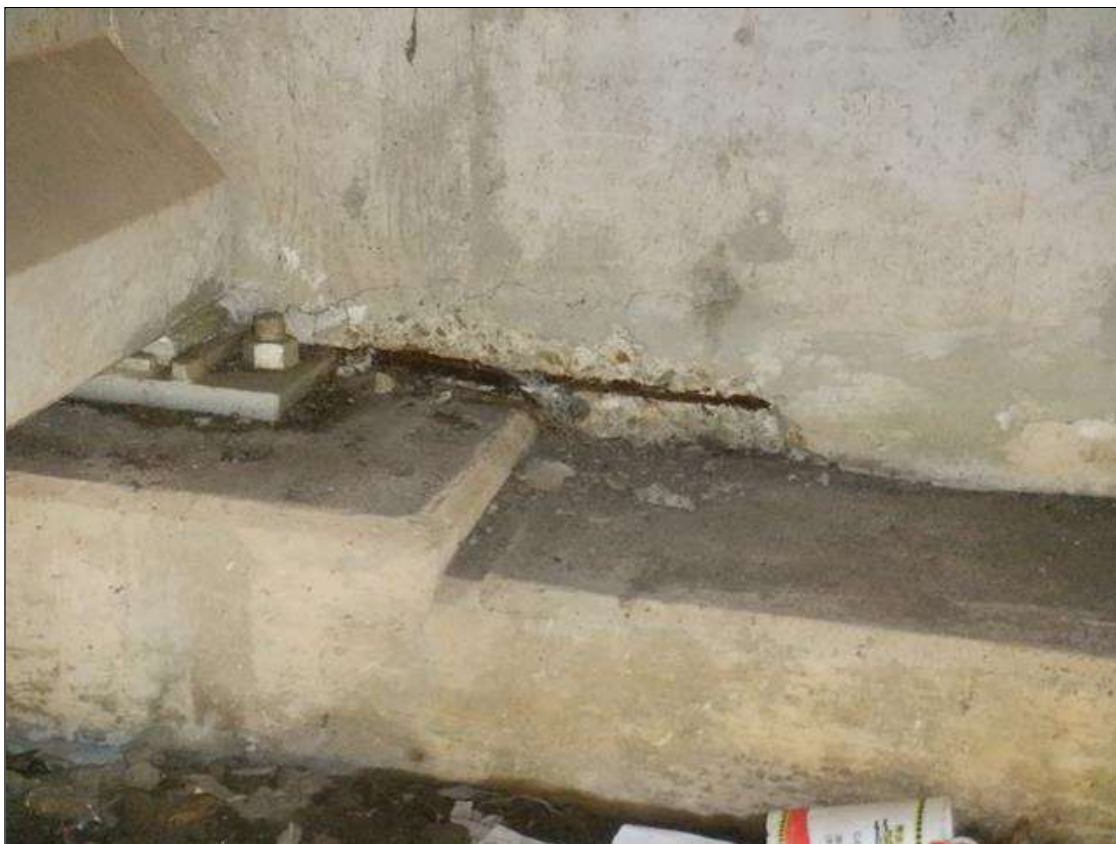
End Bent 1 Abutment: 3 FEET X UP TO 2 INCHES X 1 INCHES SPALL WITH EXPOSED REINFORCING ON NORTH FACE BETWEEN BEAMS 1 AND 2.
