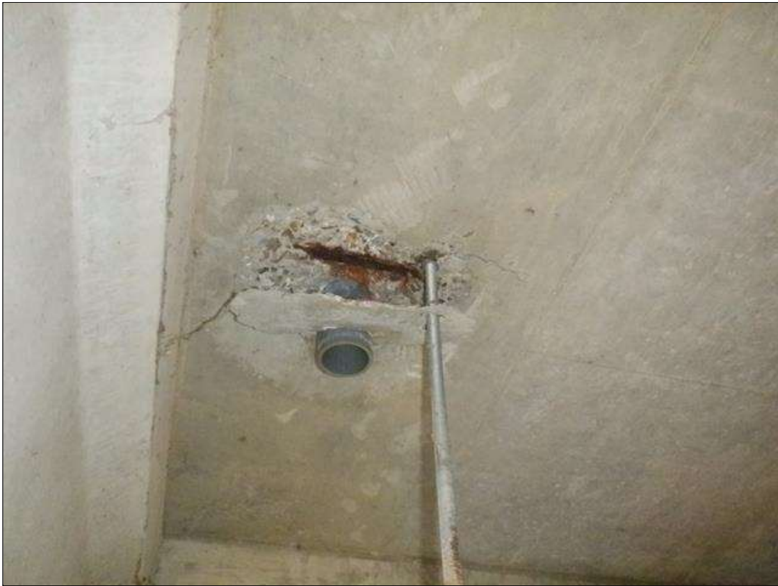
Span 3 Deck: 2 FEET X UP TO 1 FEET X 1 INCHES SPALL WITH EXPOSED REINFORCING ON DECK UNDERSIDE AROUND THIRD DRAIN BETWEEN BEAMS 7 AND 8 MEASURED FROM BENT 3.
