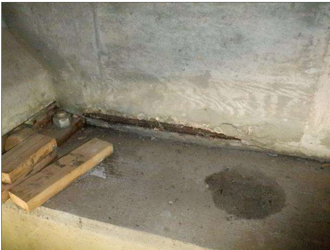
End Bent 1 Abutment: 27 INCHES X UP TO 4 INCHES X 1 INCHES SPALL WITH EXPOSED REINFORCING ON NORTH FACE BETWEEN BEAMS 6 AND 7.
