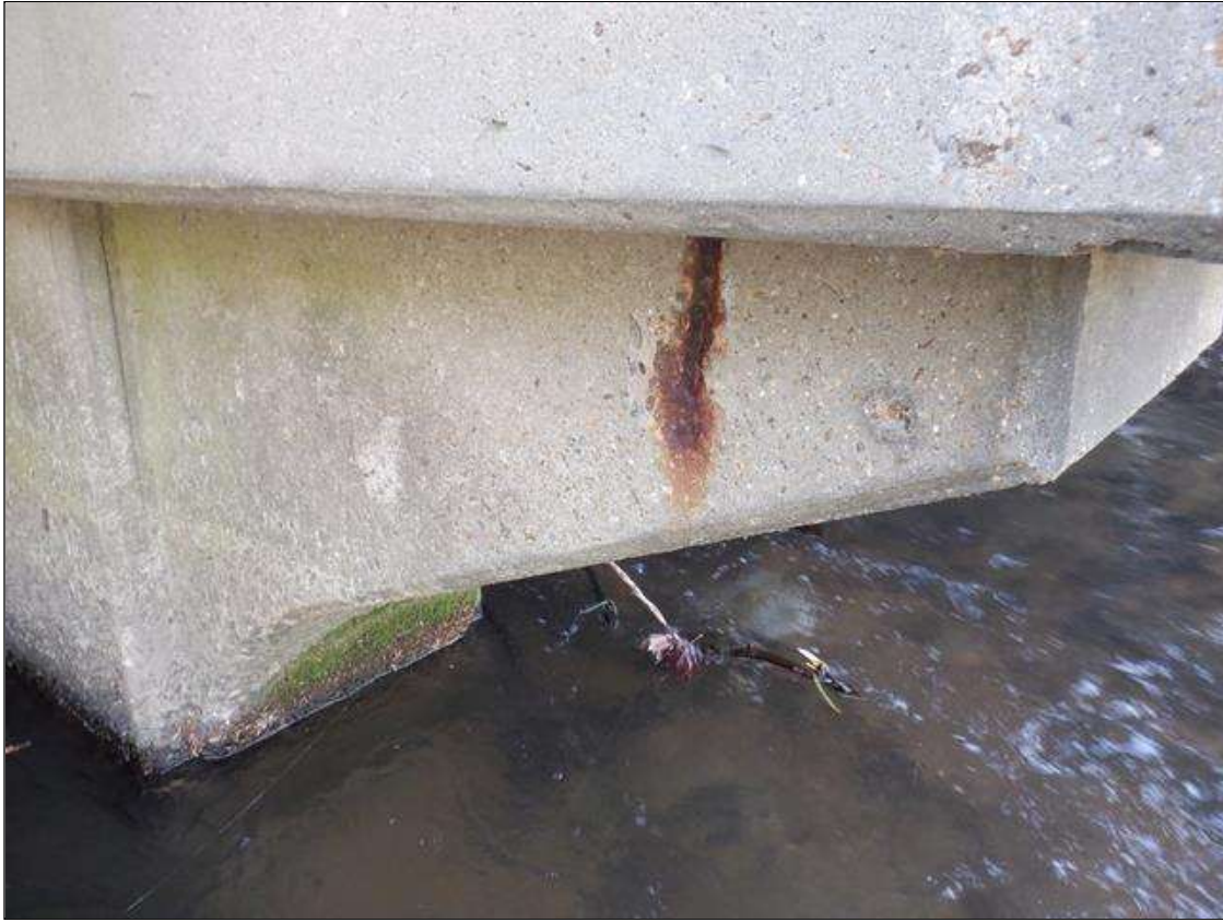
Bent 3 Cap 1: 2 INCHES X UP TO 6 INCHES X 1 INCHES SPALL WITH EXPOSED REINFORCING ON SOUTH FACE OF EAST OVERHANG.
