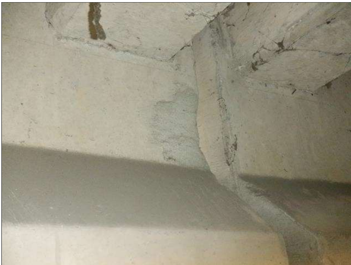
Span 2 Beam 4: 4 INCHES X UP TO 8 INCHES PATCHED AREA ON EAST FACE OF WEB AT BENT 2.
