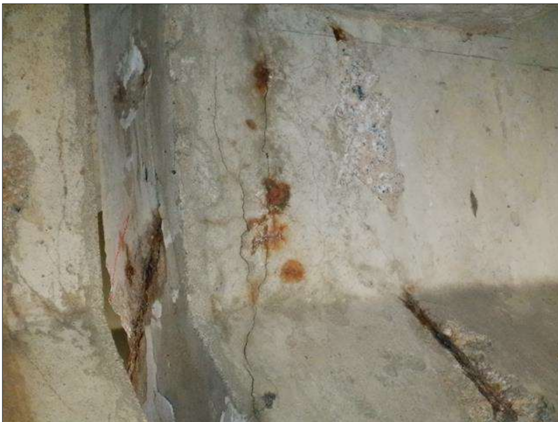
Span 2 Beam 6: (PAR) 5 INCHES X UP TO 11 INCHES AREA OF UP TO 0.014 INCHES MAP CRACKING WITH RUST STAINING ON THE WEST FACE OF THE WEB AND CHAMFER AT BENT 2.
