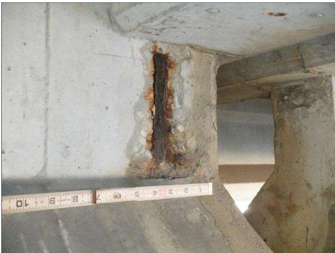
Span 1 Beam 6: 5 INCHES X UP TO 8 INCHES X 1/4 INCHES SPALL WITH EXPOSED REINFORCING ON EAST FACE AT BENT 1.
