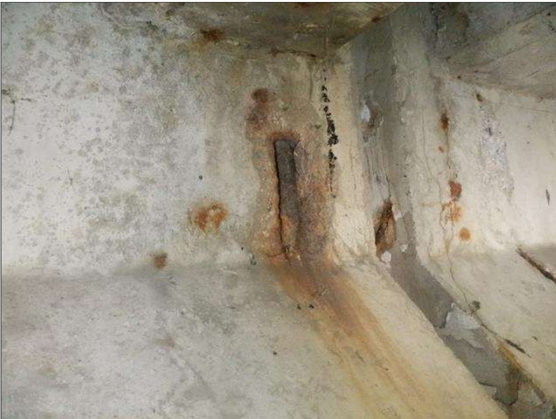
Span 3 Beam 6: (2) UP TO 4 INCHES X 7 INCHES X 1 INCHES SPALLS WITH EXPOSED REINFORCING ON EAST AND WEST FACES AT BENT 2.
