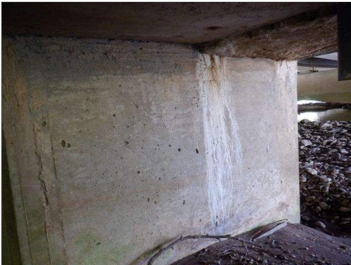
Bent 1 Pile 6: 14 INCHES X UP TO 1/64 INCHES VERTICAL CRACKS WITH EFFLORESCENCE AND HEAVY BUILDUP AT RANDOM, EXTENDING FROM BOTTOM OF CAP.
