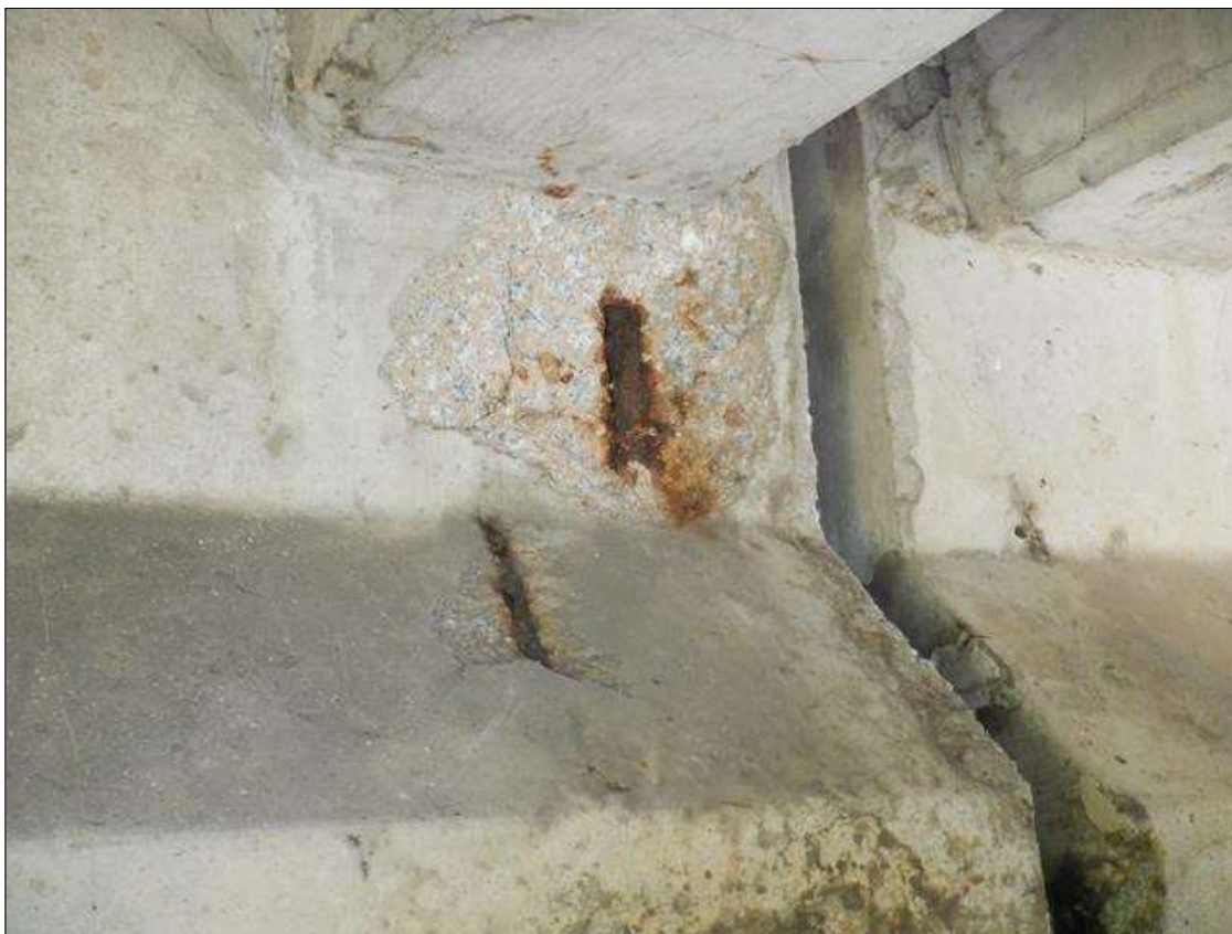
Span 4 Beam 2: (2) UP TO 10 INCHES DIAMETER X 1 INCHES SPALLS WITH EXPOSED REINFORCING ON WEST FACE AT BENT 3.
