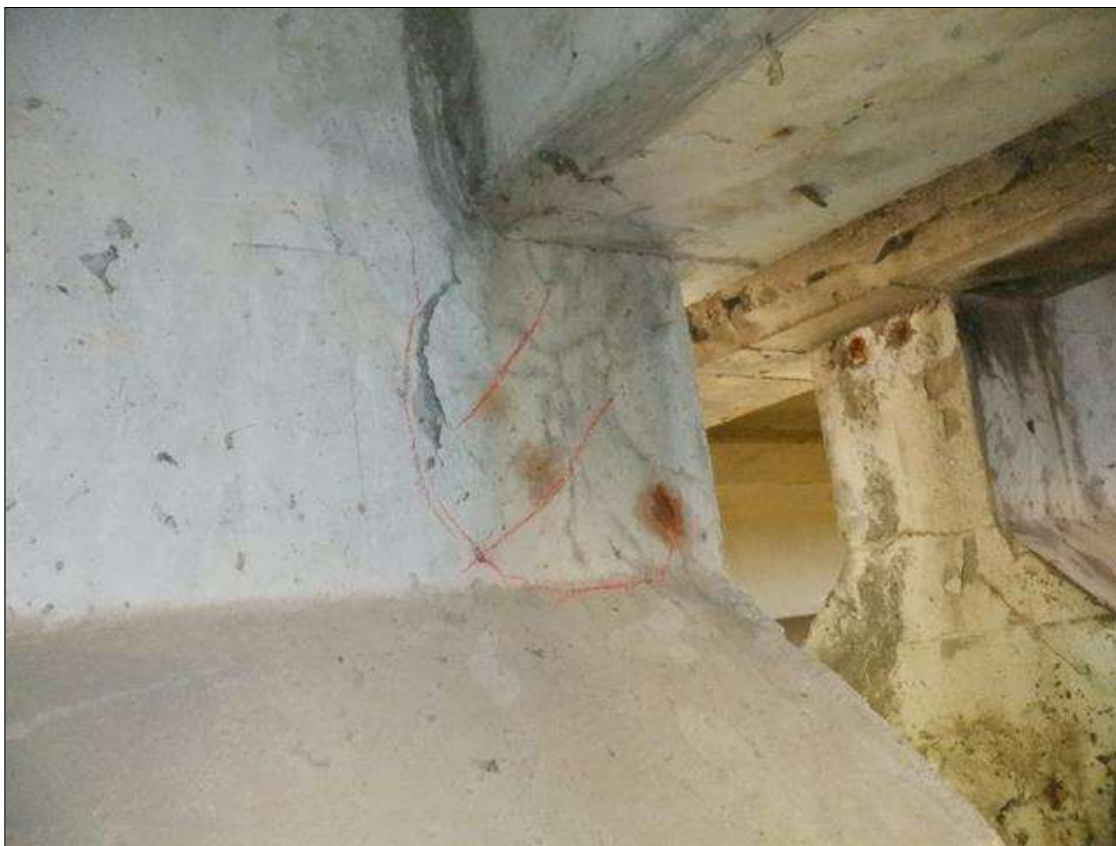
Span 1 Beam 3: 6 INCHES X UP TO 8 INCHES DELAMINATION WITH HAIRLINE MAP CRACKING AND RUST STAINING ON EAST FACE AT BENT 1.
