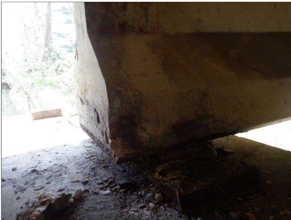
Span 2 Beam 1: 4 INCHES X 7 INCHES UP TO 1.5 INCHES SPALL WITH EXPOSED REINFORCING IN SOUTHEAST CORNER OF BOTTOM FLANGE AT BENT 1.
