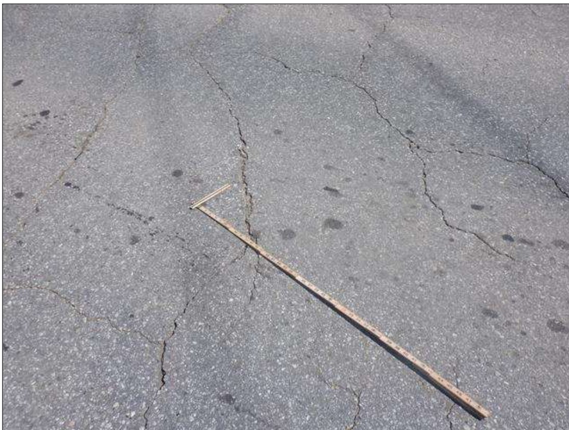
THROUGHOUT BOTH APPROACHES, MULTIPLE TRANSVERSE AND LONGITUDINAL CRACKS (8 FEET X UP TO 1/2 INCH) AND AREAS OF BROKEN AND MISSING ASPHALT
