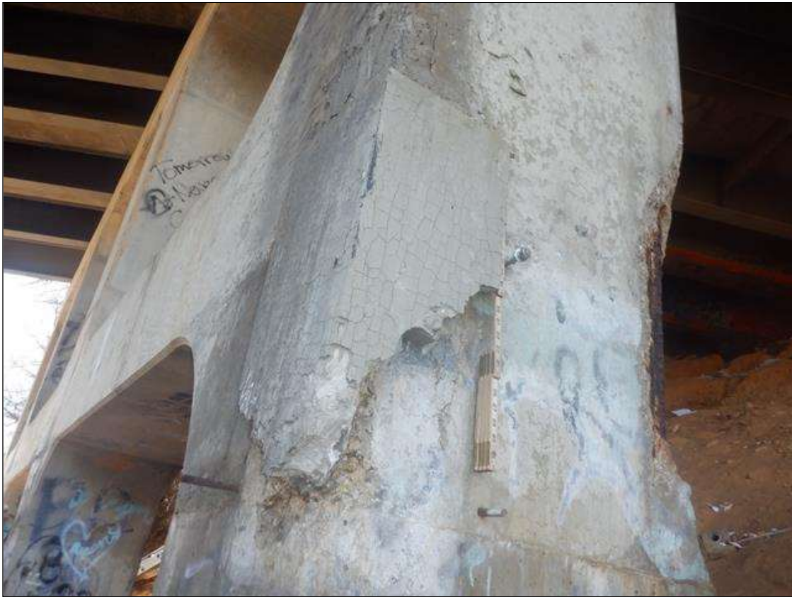
Bent 2 Pile 4: 13 FEET FROM BOTOM OF CAP AT SOUTHEAST CORNER, 2.25 FEET X 1 FEET X 2 INCHES DEEP UNSOUND CONCRETE. SPALL BENEATH PATCH WITH ASSOCIATED DELAMINATION (4 FEET X 20 INCHES)
