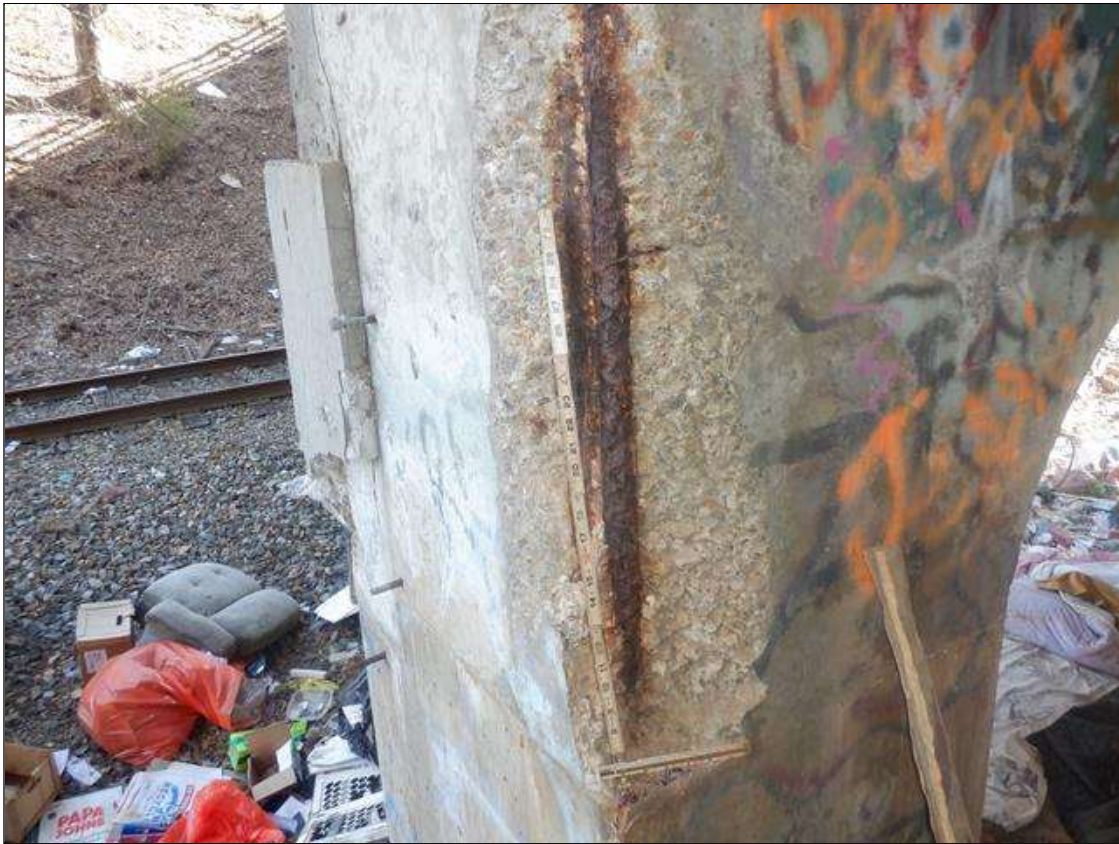
Bent 2 Pile 4: (PAR) 13 FEET FROM BOTTOM OF CAP AT NORTHEAST CORNER, 4 FEET TALL X 13 INCHES WIDE X 3 INCHES DEEP SPALL WITH EXPOSED REBAR, 10 PERCENT SECTION LOSS
