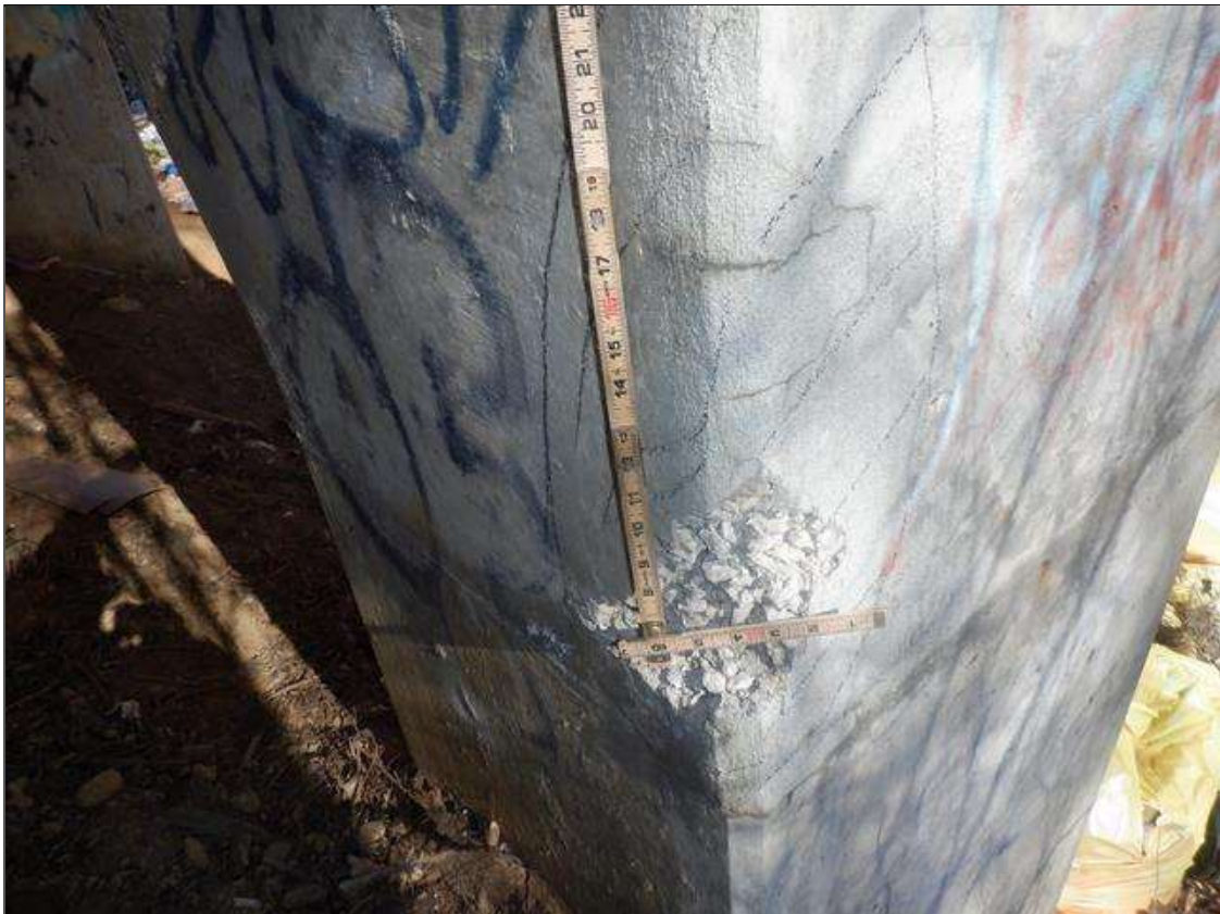
Bent 2 Pile 1: NORTHWEST CORNER, 3 FEET FROM GROUND, UNSOUND PATCH (2 FEET X 1 FEET) WITH ASSOCIATED SPALL (7 INCH DIAMETER X 2 INCH DEEP) NO EXPOSED REINFORCING
