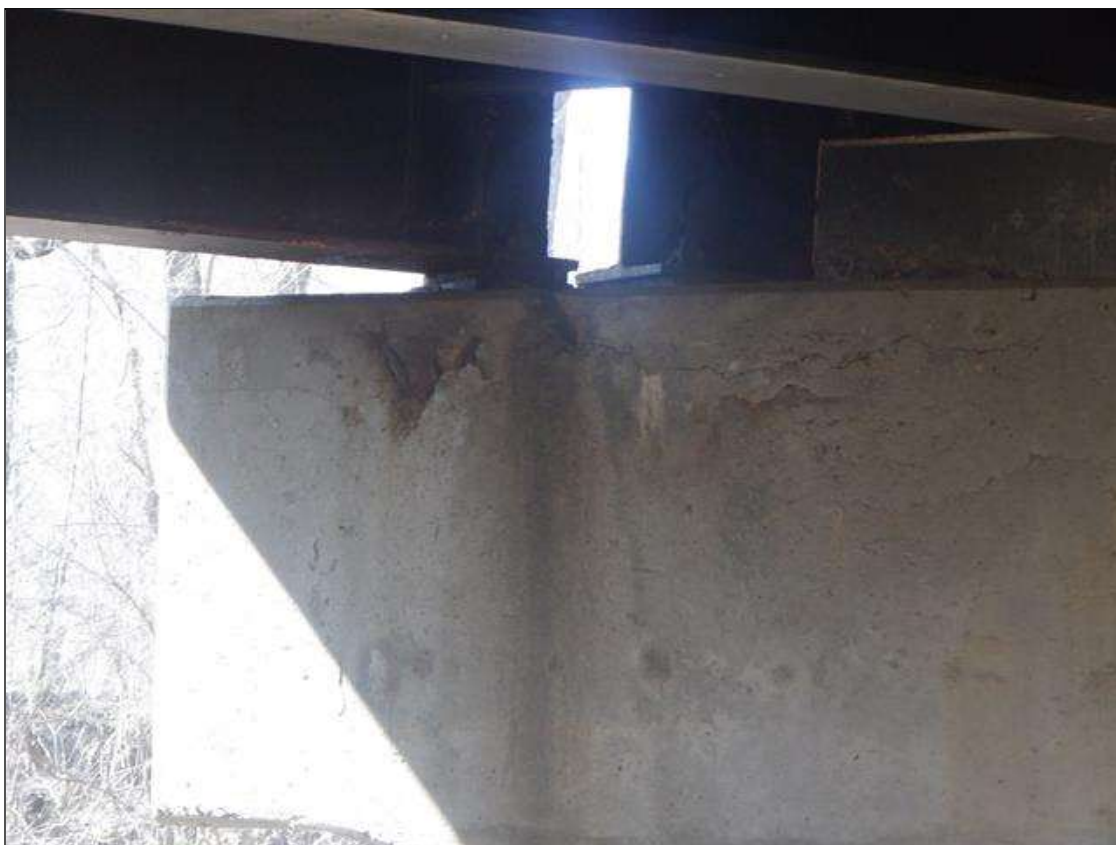
Bent 1 Cap 1: SOUTH FACE BELOW BEAM 1, 12 INCHES X UP TO 12 INCHES X 3/4 INCHES SPALL WITH EXPOSED REBAR. NO SECTION LOSS
