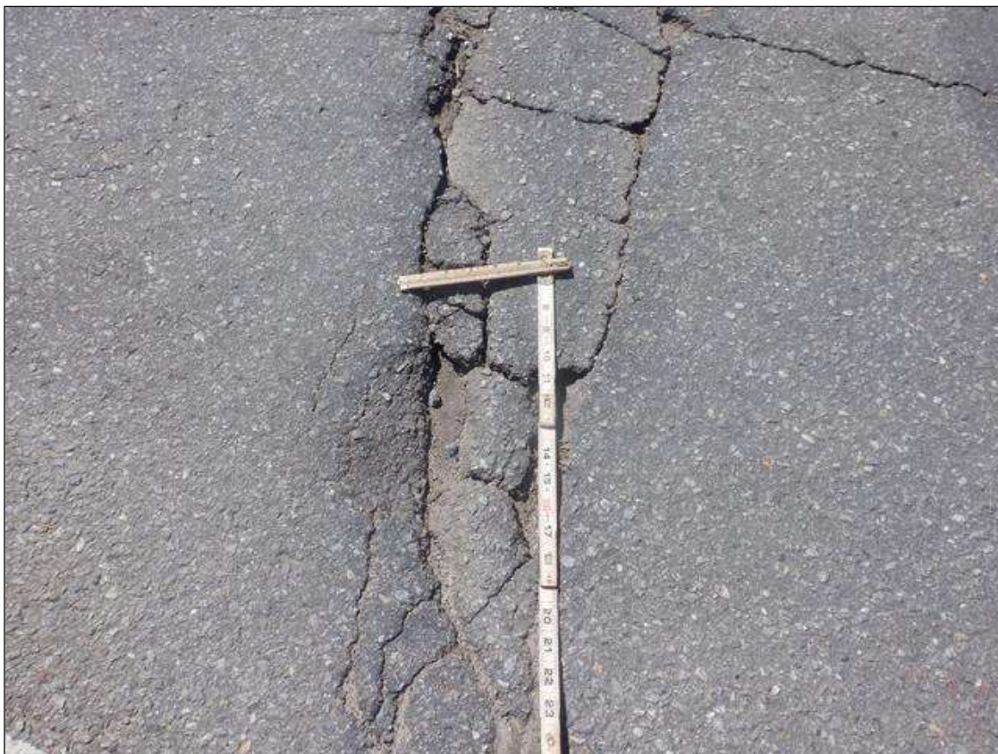
Span 3 Wearing Surface: AT END BENT 2, FULL LENGTH CRACK UP TO 1 INCHES WIDE WITH AREAS OF BROKEN AND MISSING ASPHALT
