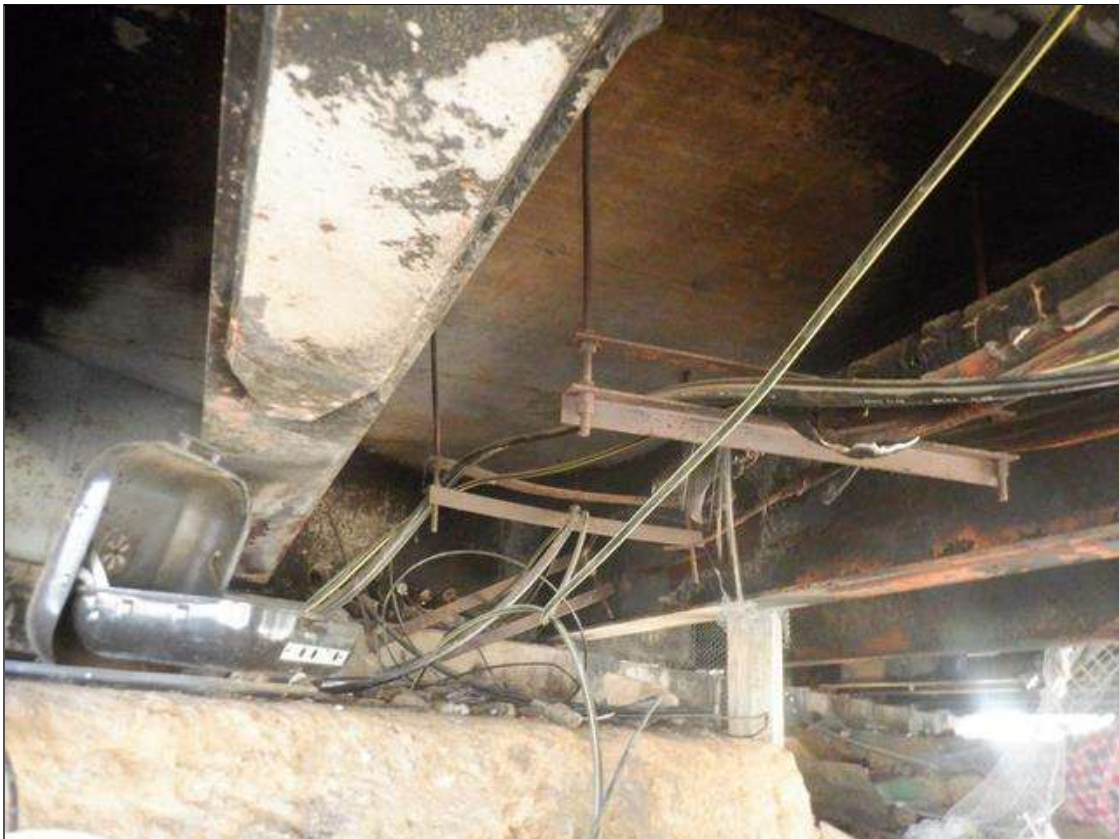
BAY 7 NINE (9) 4 INCH DIAMETER UTILITIES, BROKEN FROM FIRE DAMAGE
