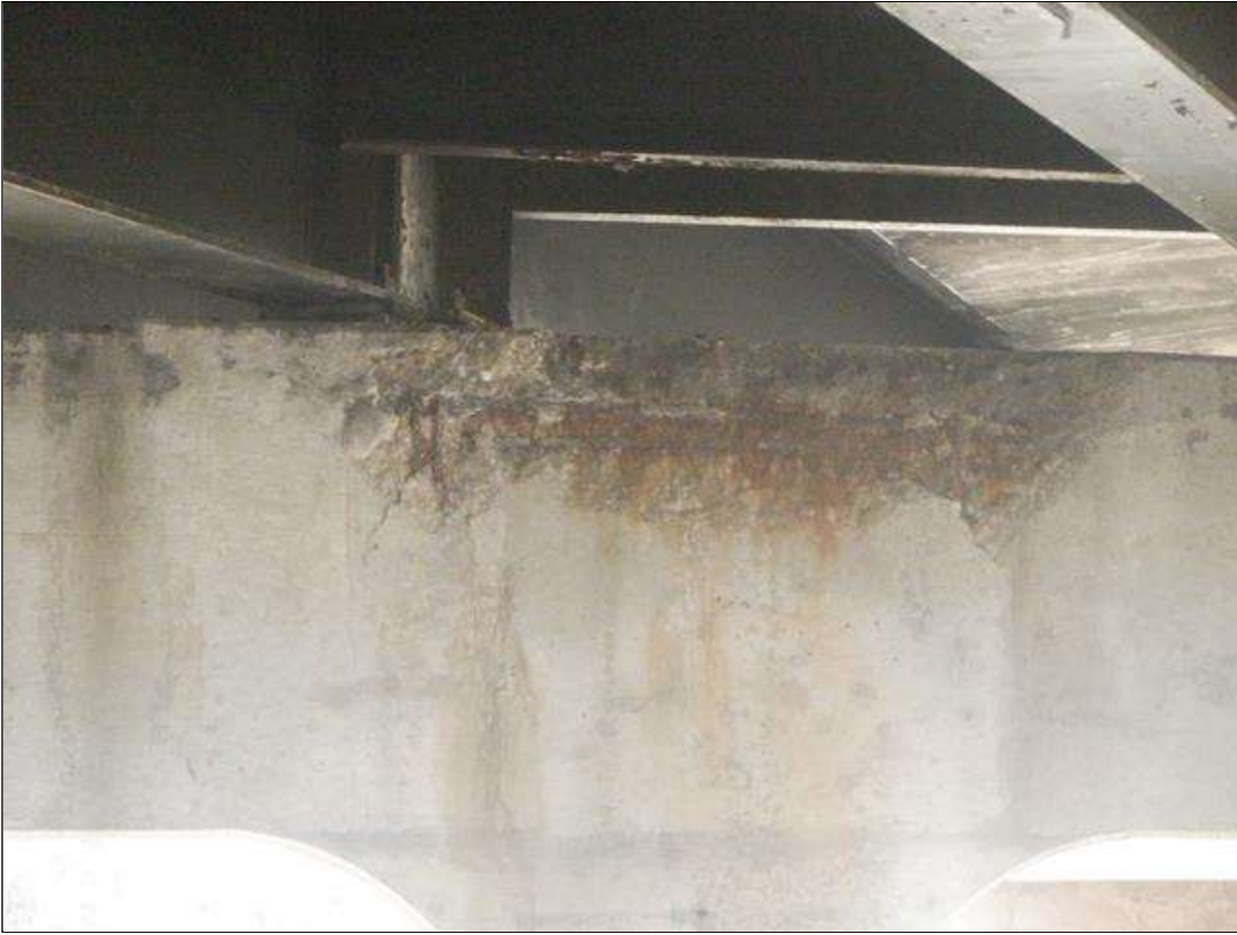
Bent 1 Cap 1: (PAR) TOP AND SOUTH FACES BELOW BEAM 3 AND 4, 5.5 FEET X UP TO 18 INCHES X 5 INCHES DEEP SPALL WITH EXPOSED REBAR WITH 10 PERCENT SECTION LOSS
