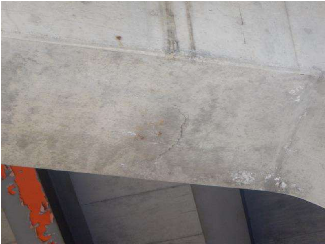
Bent 2 Cap 1: SOFFIT BETWEEN PILES 2 AND 3, 9 INCHES LONG DELAMINATION (SIMILAR BETWEEN PILE 1 AND PILE 2)
