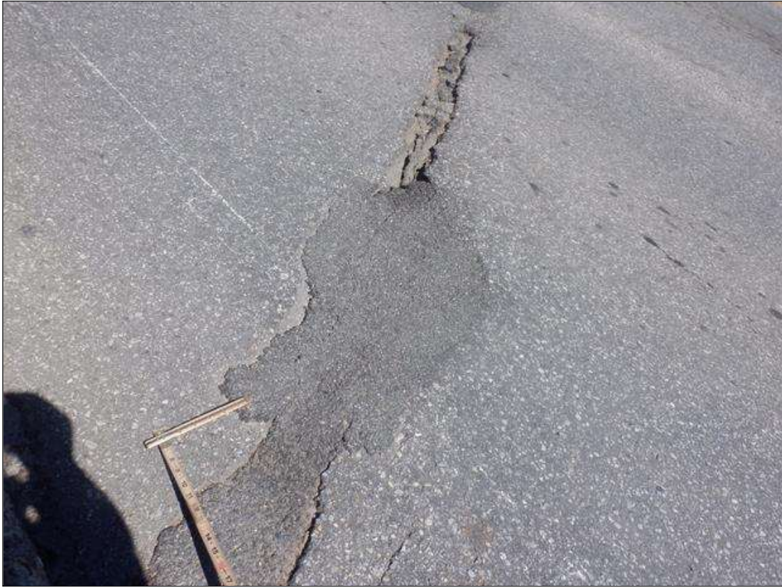
Span 2 Wearing Surface: AT BENT 1, 15 SQUARE FEET OF SOUND PATCHES SCATTERED THROUGHOUT
