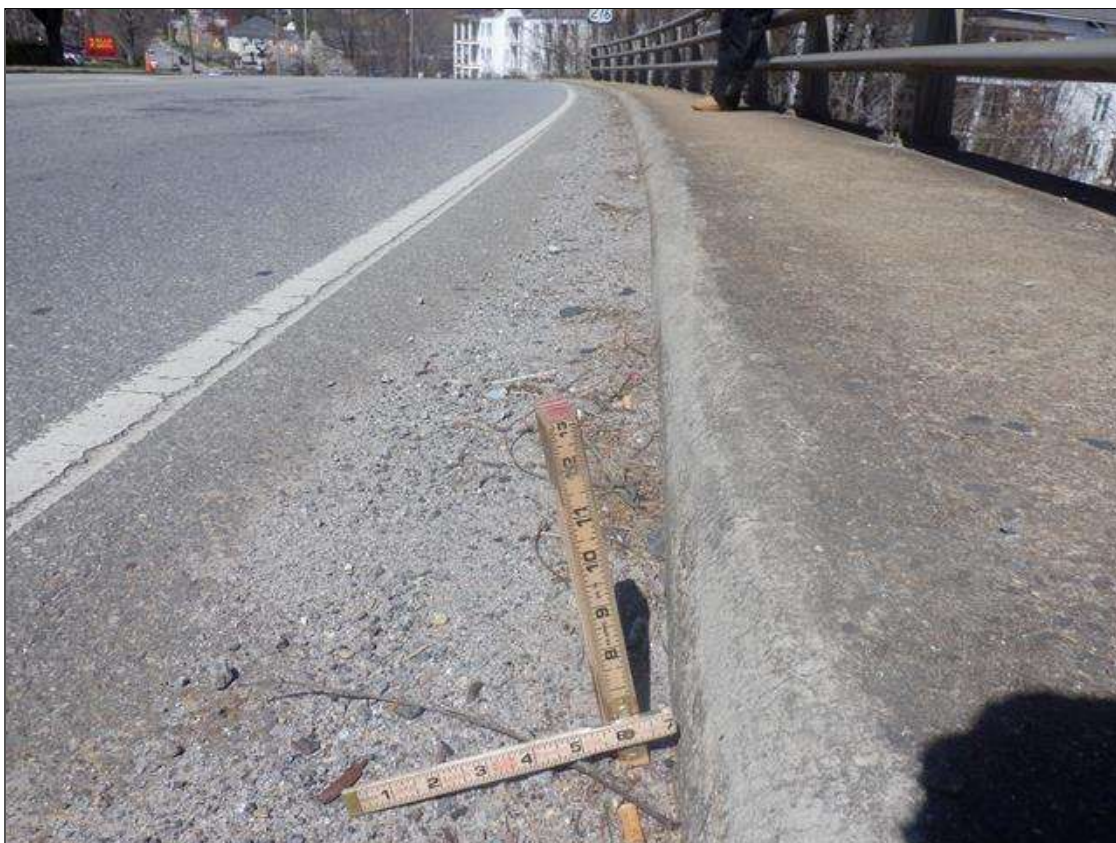
GRAVEL AND DEBRIS ALONG RIGHT CURB
