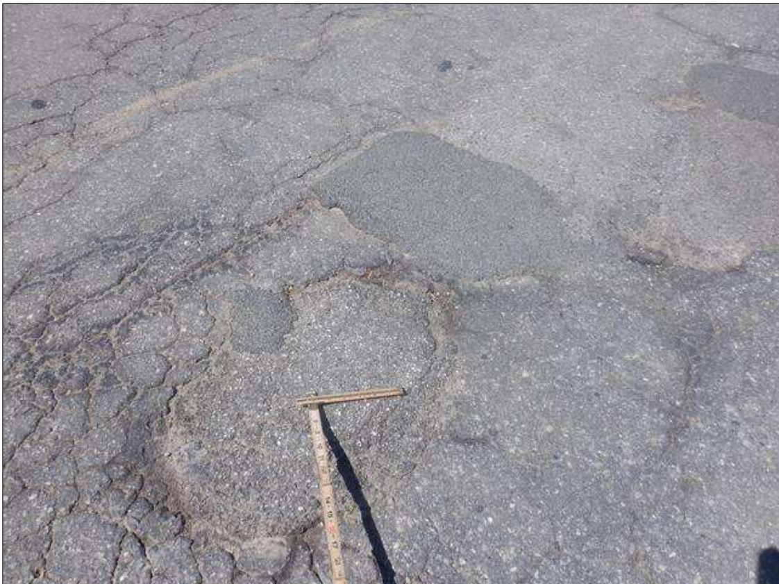
Span 2 Wearing Surface: BETWEEN NORTHBOUND LANES, 20 FEET FROM BENT 2, MULTIPLE SCATTERED SOUND PATCHES UP TO 3 FEET DIAMETER
