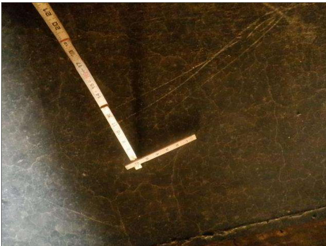
Span 1 Deck: DECK UNDERSIDE THROUGHOUT AREAS OF MAP CRACKING UP TO 1/64 INCHES
