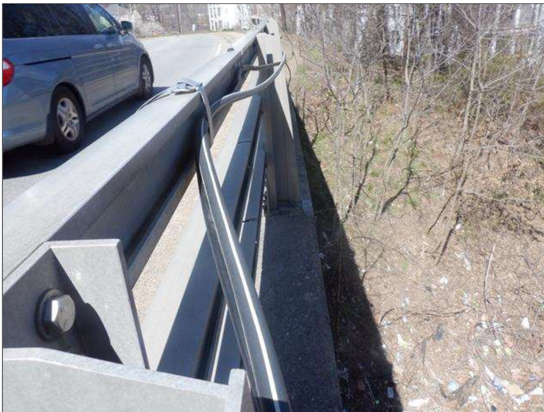
ATTACHED UTILITY AT RIGHT BRIDGE RAIL
