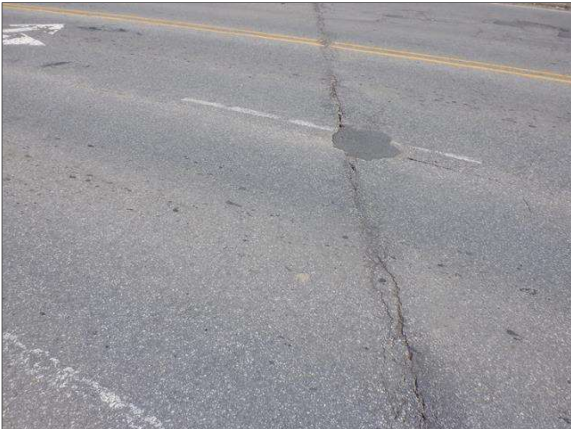
ASPHALT OVER BENT 2 (ASPHALT OVER BENT 1 SIMILAR)
