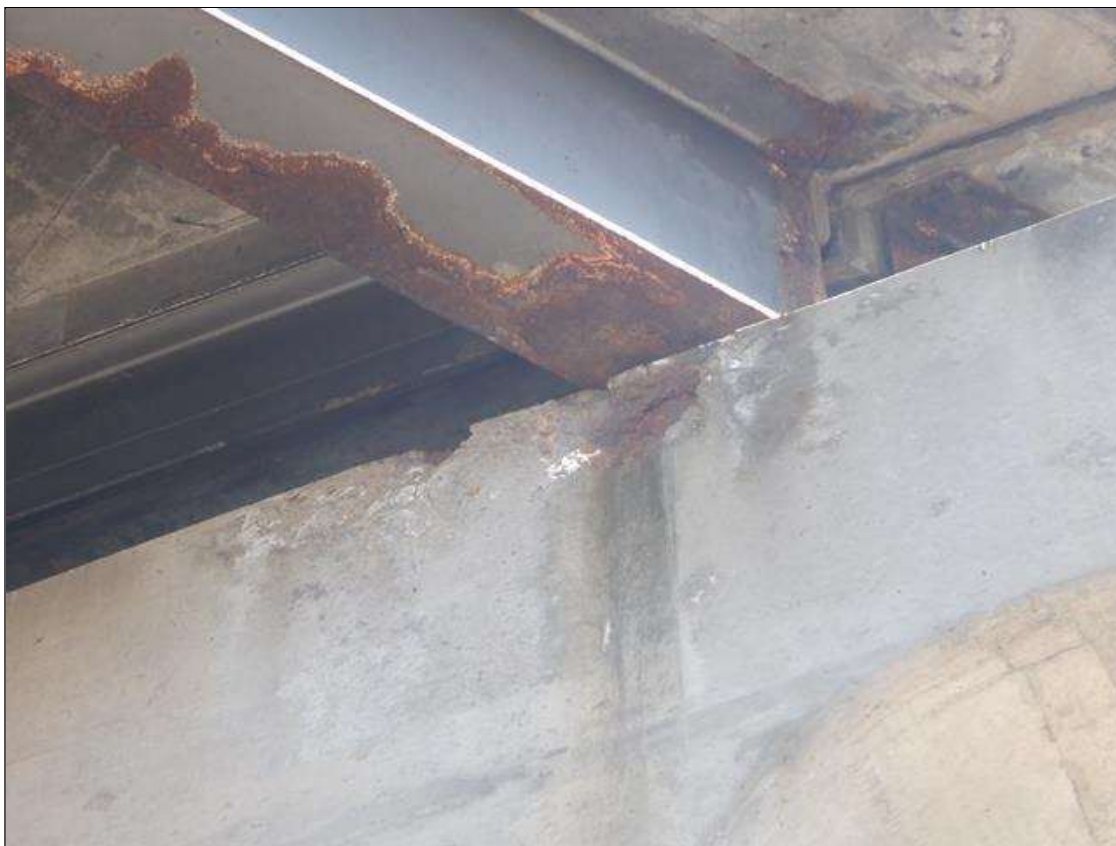
Bent 1 Cap 1: NORTH FACE AT TOP OF CAP AT BEAMS 1 AND 5, (2) UP TO 12 INCHES X 6 INCHES X 1 INCHES DEEP SPALLS
