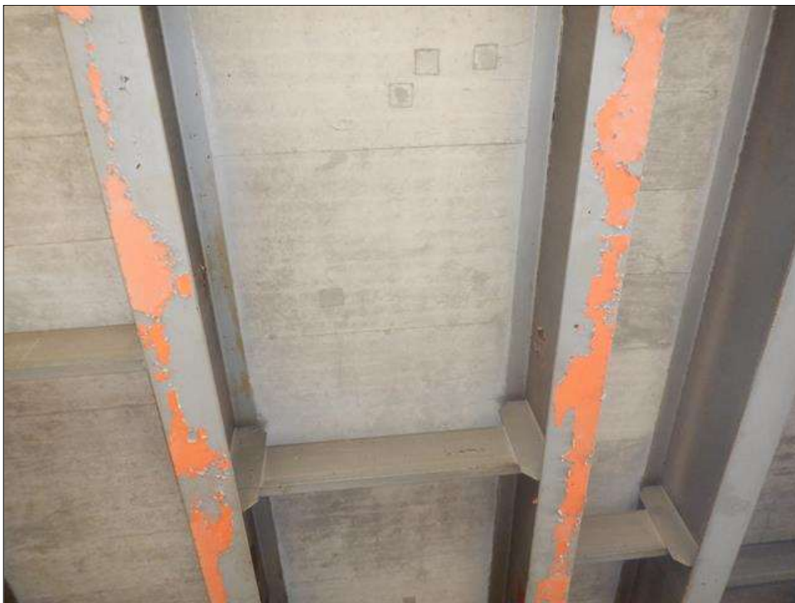
Span 3 Beam 4 - Protective System: PEELING FINISH COAT ALONG LENGTH OF BOTTOM FLANGE
