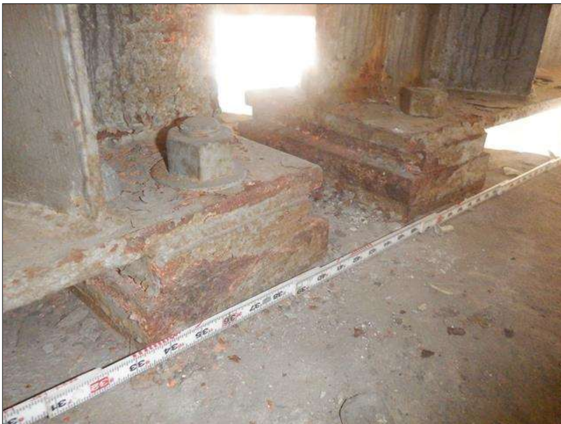
Span 3 Near Bearing: SURFACE CORROSION THROUGHOUT BEARING
