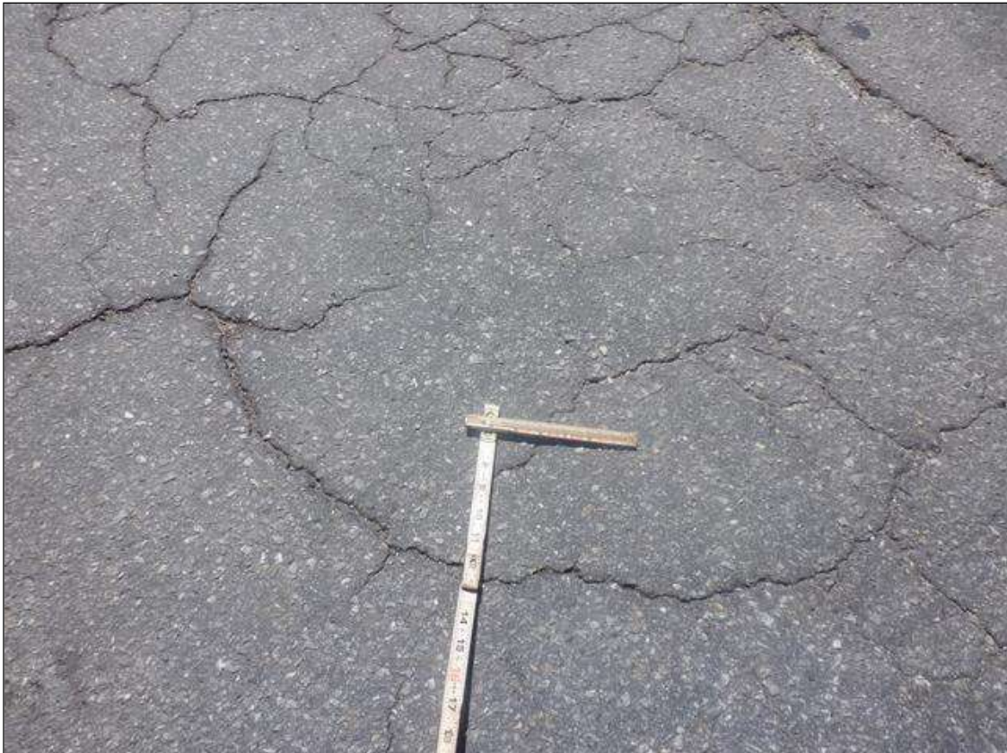
Span 2 Wearing Surface: THROUGHOUT NORTHBOUND LANES, MAP CRACKING UP TO 1/8 INCHES WIDE
