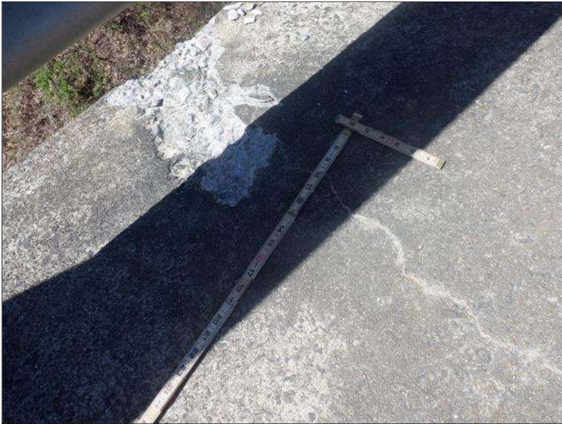
Span 2 Left Bridge Rail: SIDEWALK NEAR MID SPAN, HAIRLINE TRANSVERSE CRACK WITH ADJACENT SPALL (18 INCHES X 7 INCHES X 3/4 INCHES DEEP)
