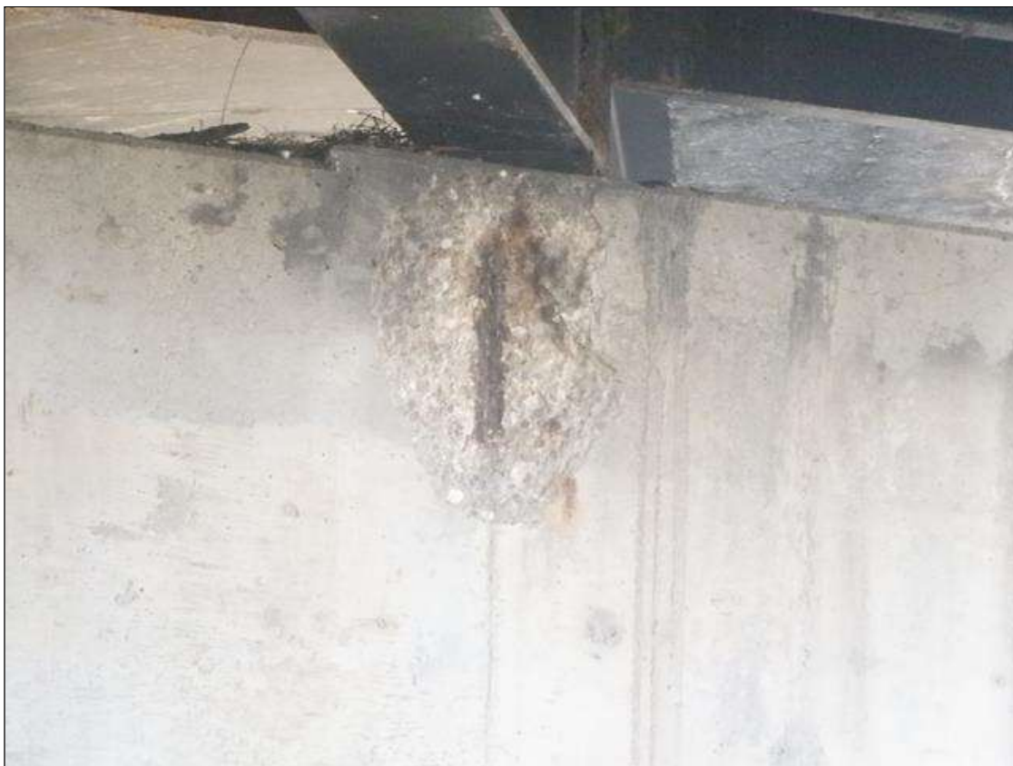
Bent 1 Cap 1: (PAR) SOUTH FACE BELOW BEAM 6, 18 INCHES X UP TO 24 INCHES X 2 INCHES DEEP SPALL WITH EXPOSED REBAR WITH 10 PERCENT SECTION LOSS
