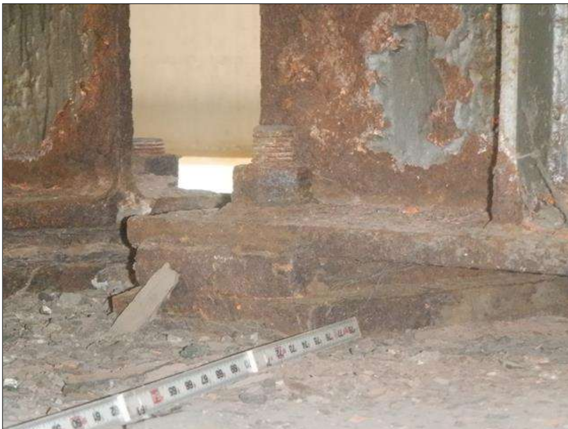
Span 3 Near Bearing: CORROSION WITH ONSET OF SECTION LOSS
