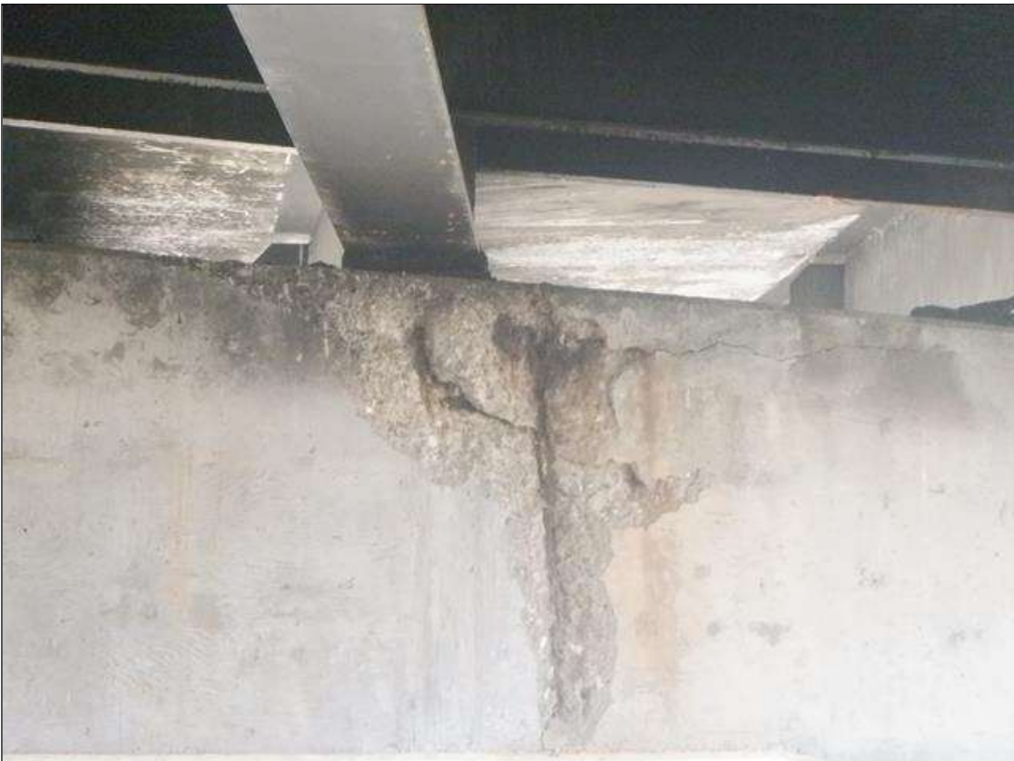
Bent 1 Cap 1: (PAR) SOUTH FACE BELOW BEAM 5, 5 FEET X UP TO 3 FEET X 3 INCHES DEEP SPALL WITH EXPOSED REBAR WITH 10 PERCENT SECTION LOSS
