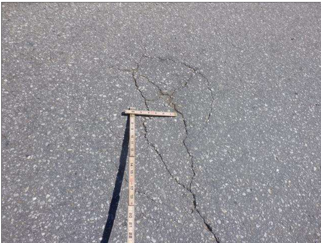
Span 2 Wearing Surface: THROUGHOUT SOUTHBOUND LANES, MAP CRACKING UP TO 1/8 INCHES WIDE SCATTERED THROUGHOUT
