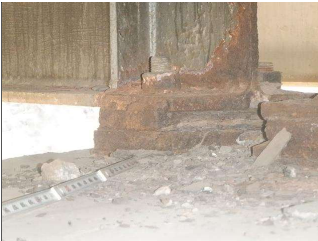
Span 2 Beam 2 - Far Bearing: CORROSION WITH ONSET OF SECTION LOSS
