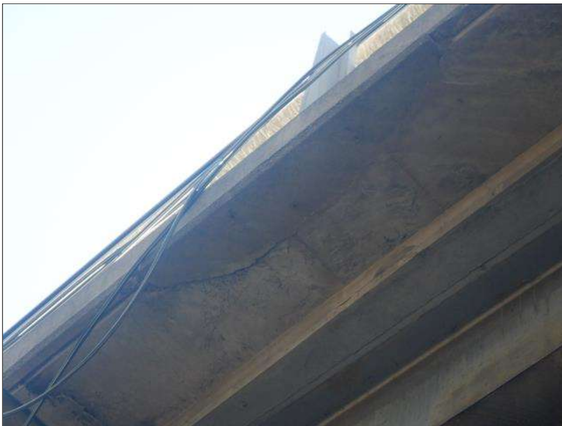
Span 2 Deck: RIGHT OVERHANG AT BENT 1, 4.5 FEET LONG X 1 FEET WIDE SOUND PATCH
