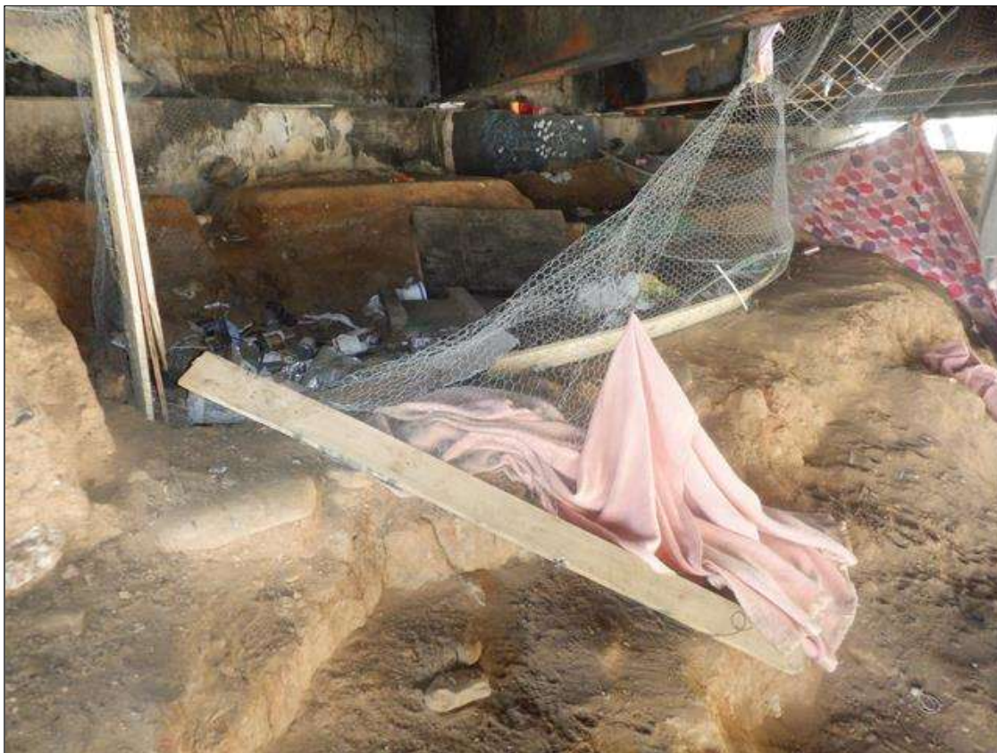
General Comments: AT BOTH END BENTS, EVIDENCE OF ACTIVE VAGRANCY
