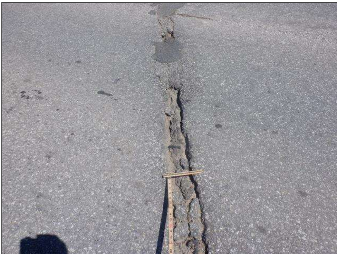
Span 2 Wearing Surface: AT BENT 1, MULTIPLE POTHOLES UP TO 3 FEET LONG X 4 INCHES WIDE X 2 INCHES DEEP
