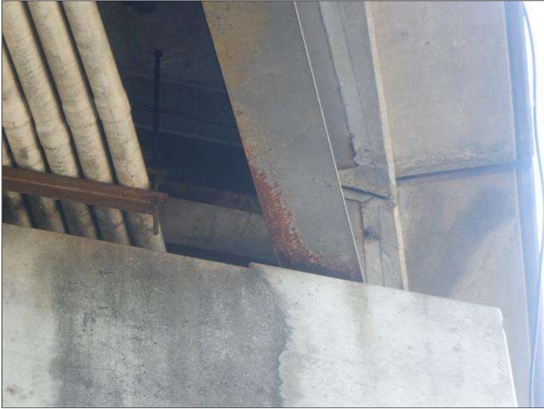
Span 2 Beam 8: AT BENT 1, 1 FEET LIGHT SCALING BOTTOM FLANGE AND UP TO 24 INCHES IN THE WEB
