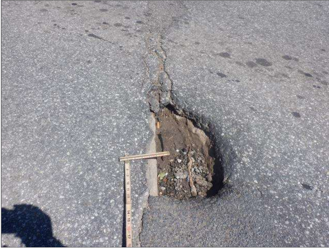
Span 2 Wearing Surface: (PAR) IN SOUTHBOUND LANE 7 FEET FROM CENTER LINE, FAILED PATCH/POTHOLE (20 INCHES X 11 INCHES X 5 INCHES DEEP)
