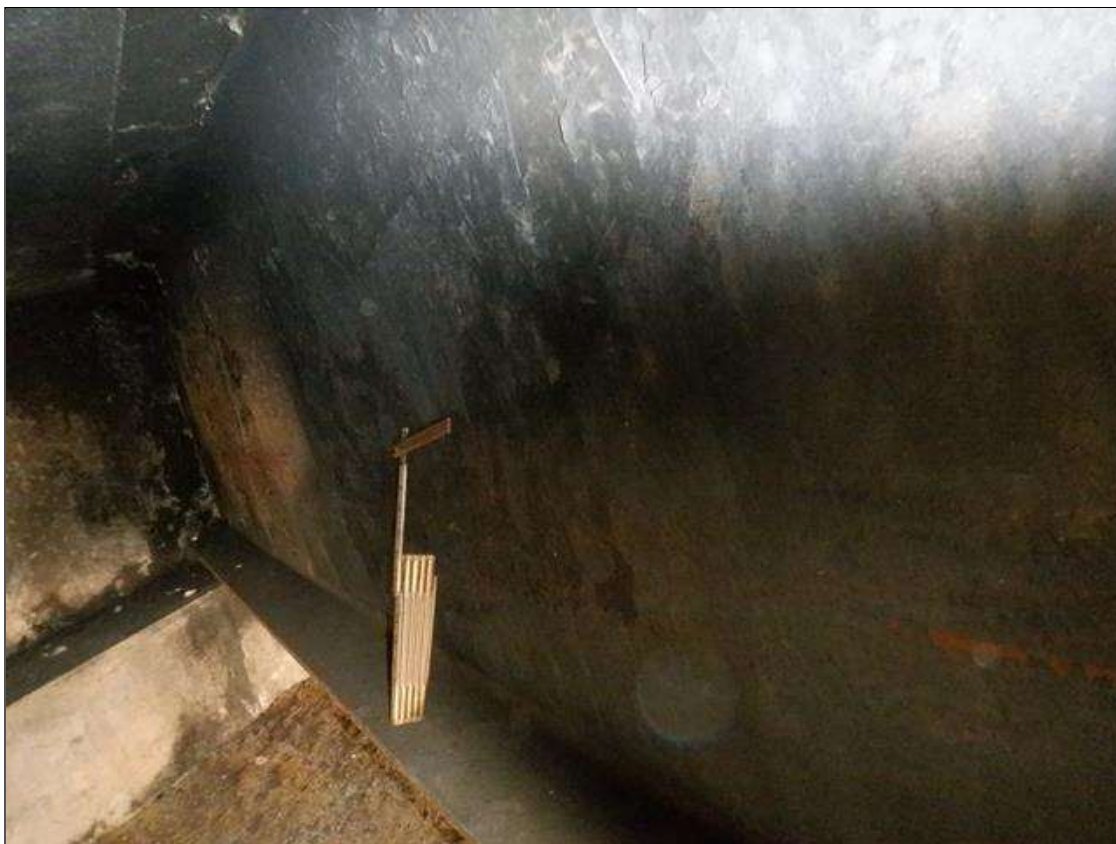
Span 1 Beam 2: 5 FEET OF BEAM / FIRE DAMAGE, 1/4 INCHES EASTWARD BULGING IN THE WEB 2 FEET FROM END BENT 1.
