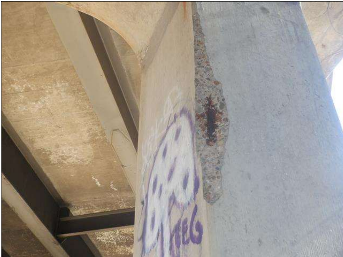
Bent 2 Pile 1: (PAR) 4 FEET FROM BOTTOM OF CAP AT NORTHEAST CORNER, 4 FEET HIGH X 3 INCHES WIDE X 3 INCHES DEEP SPALL WITH EXPOSED REBAR WITH 5 PERCENT SECTION LOSS
