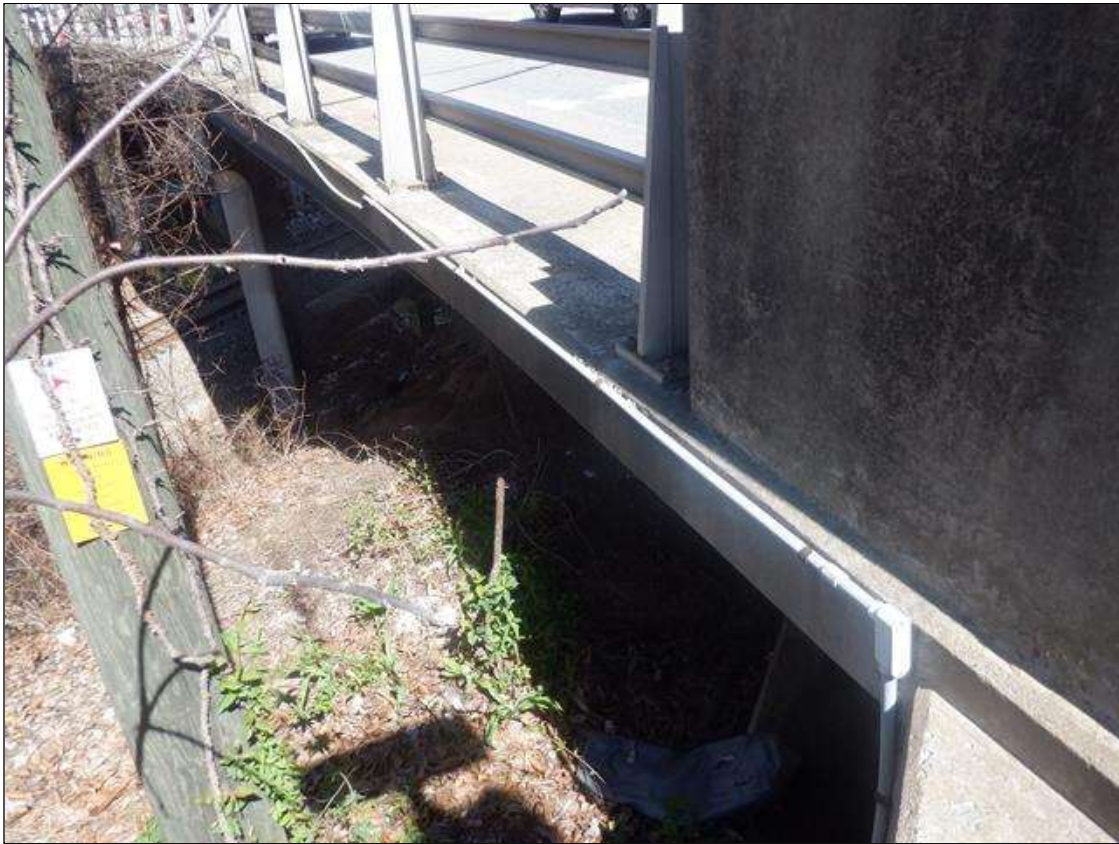
ATTACHED UTILITY AT LEFT BRIDGE RAIL (PVC CONDUIT)
