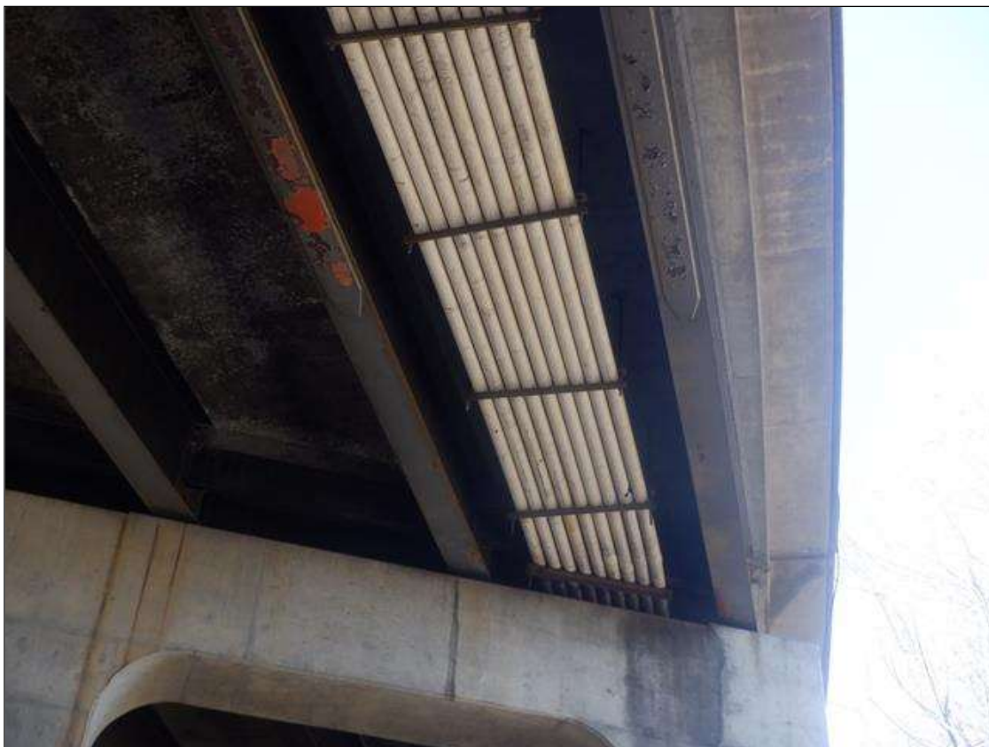
ATTACHED UTILITY AT BAY 7 (NINE (9) PVC CONDUITS)
