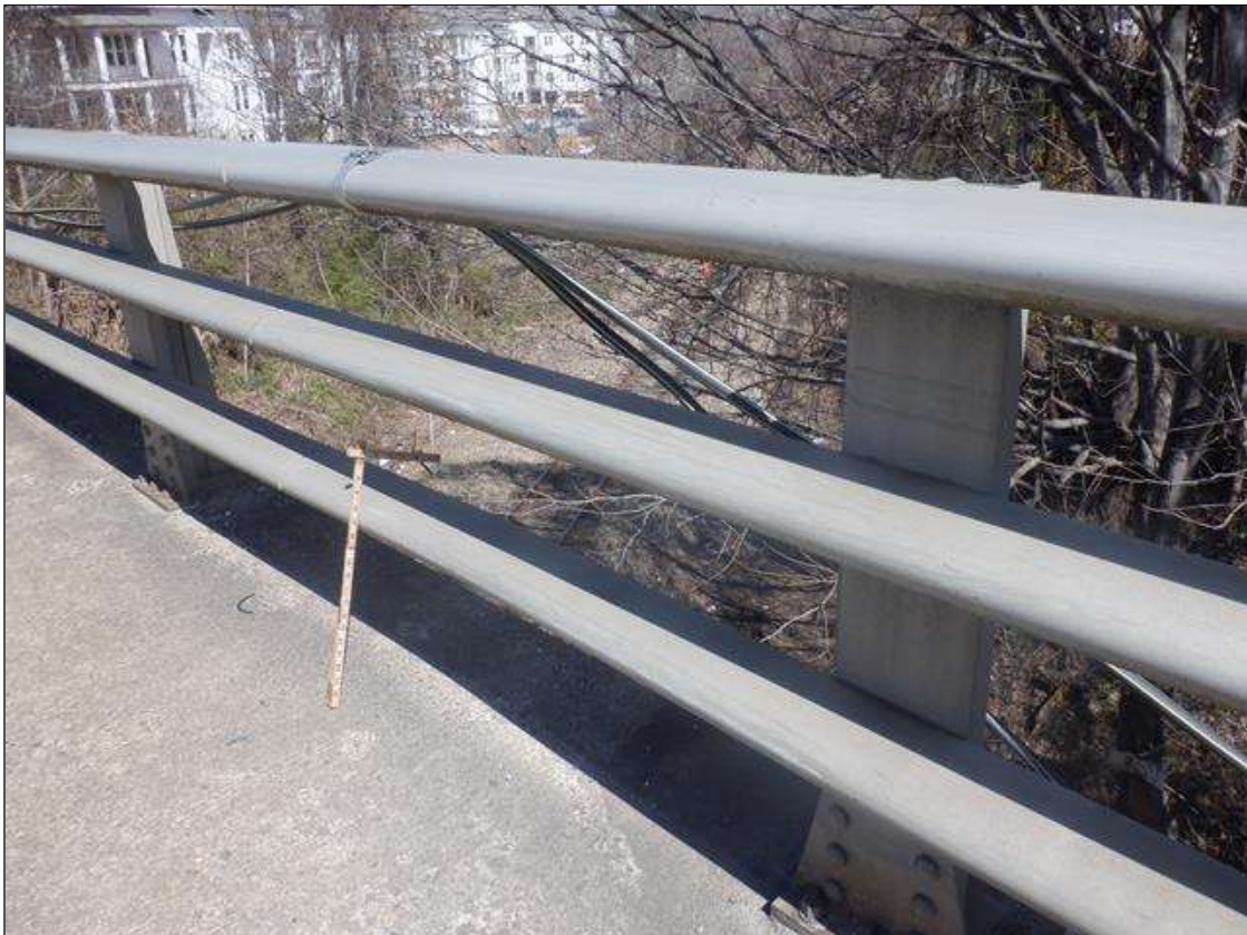
Span 2 Right Bridge Rail: STARTING AT BENT 1, VEHICULAR IMPACT DAMAGE (4 FEET LONG X 2 INCH DEFLECTION)
