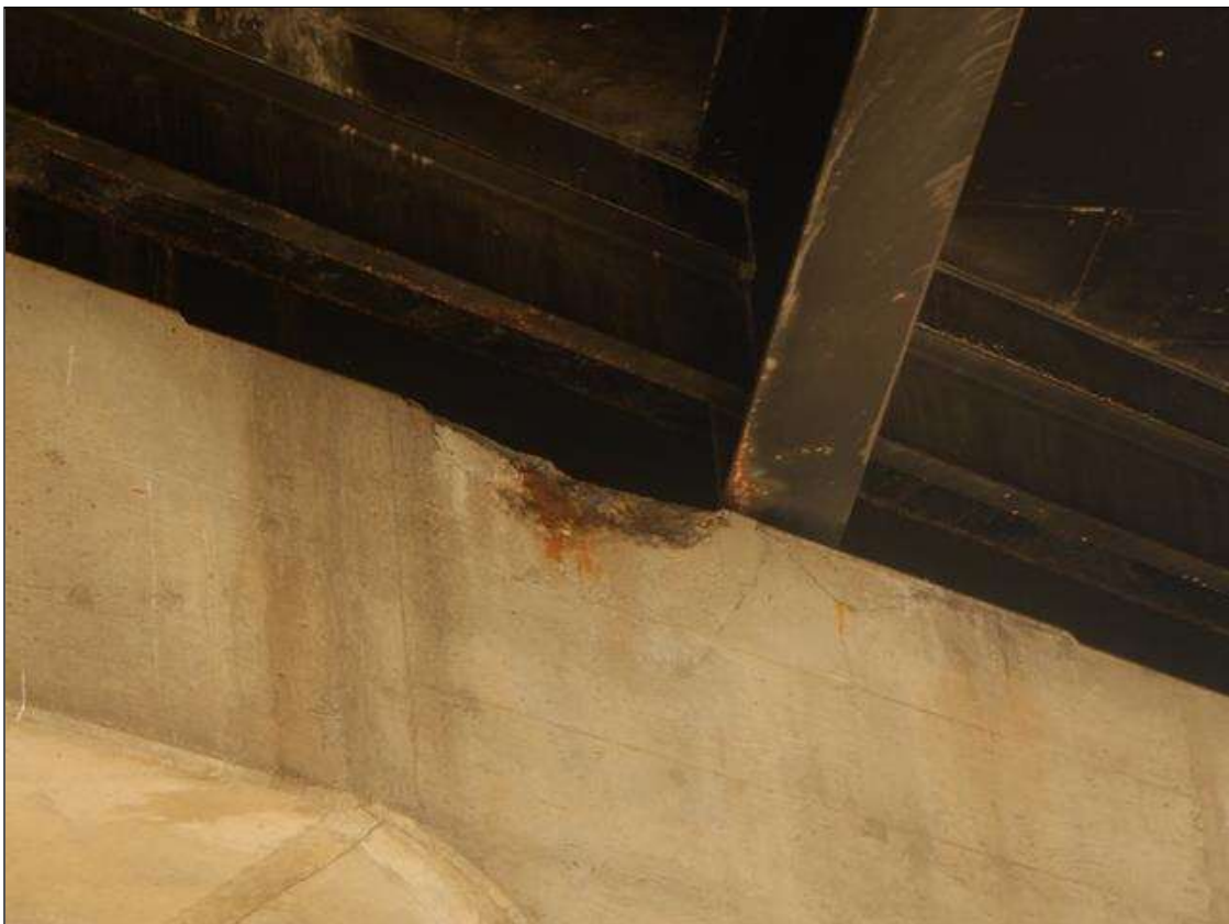
Bent 1 Cap 1: (PAR) NORTH FACE AT TOP OF CAP AT BEAM 3, 2 FEET X UP TO 1 FOOT X 1 INCHES DEEP SPAL WITH EXPOSED REBAR WITH 5 PERCENT SECTION LOSS
