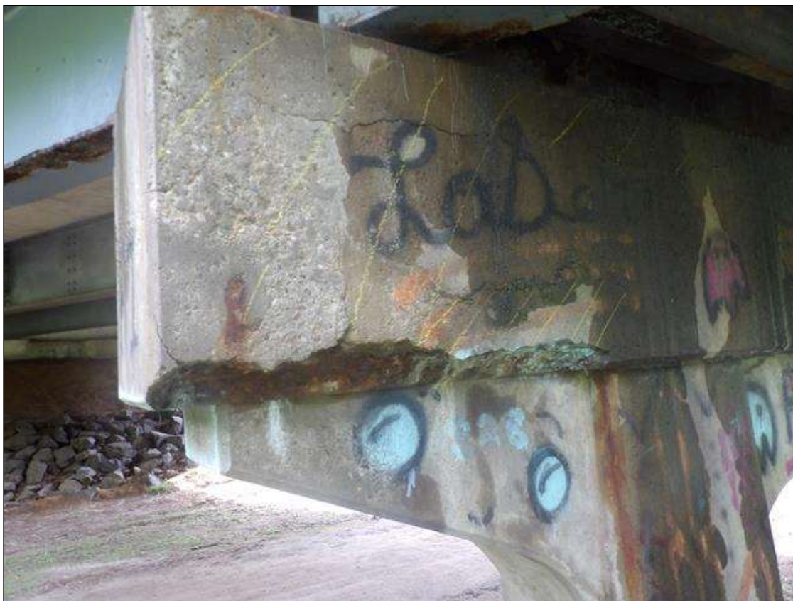
Bent 3 Cap 1: PAR: 78 INCHES X 30 INCHES X 9 INCHES AREA OF DELAMINATION WITH UP TO 1/16 INCHES VERTICAL AND HORIZONTAL CRACKS AND 48 INCHES X 6 INCHES X 6 INCHES SPALL WITH EXPOSED REBAR WITH MINOR SECTION LOSS IN TOP, BOTTOM, LEFT END AND SPAN 3 FACE OF CAP
