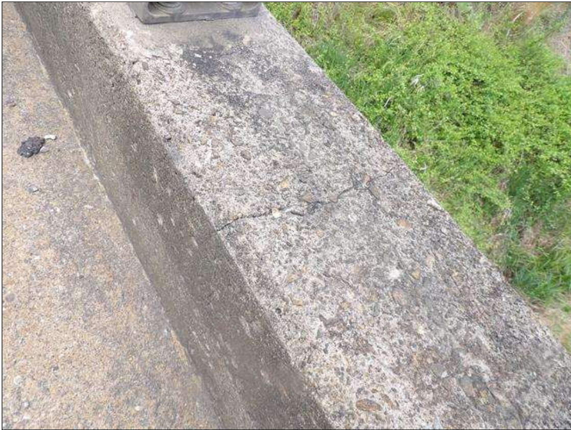
TYPICAL UP UP TO 1/32 INCHES TRANSVERSE AND VERTICAL CRACKS SCATTERED THROUGHOUT
