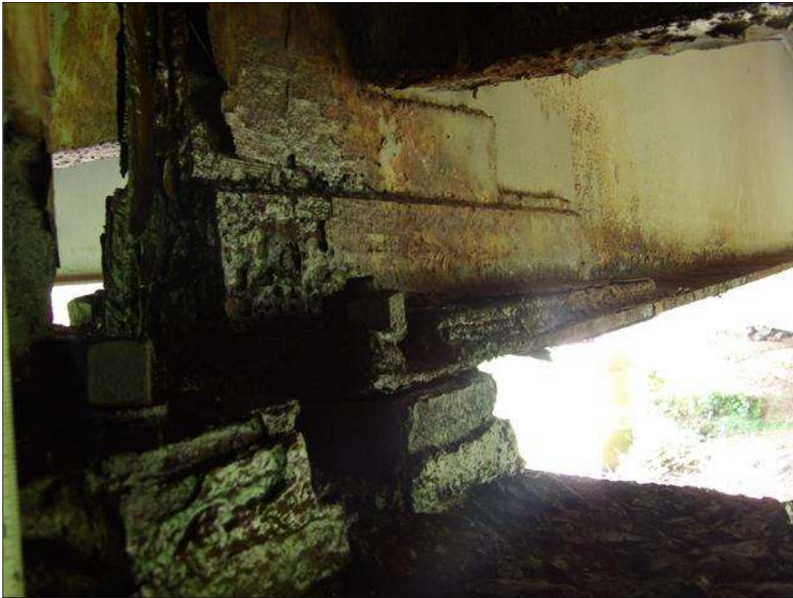
SPAN 2 BEAM 2 AT BENT 2, WELDED PLATE REPAIRS ON BOTH FACES OF WEB AND BOTTOM FLANGE UP TO 36 INCHES LONG X 20 INCHES HIGH 1/2 INCH THICK IN WEB, AND 36 INCHES LONG X 4 INCHES WIDE X 4 INCH HIGH X 1/2 INCH THICK ANGLE
