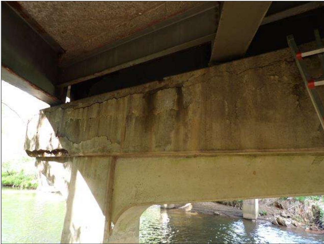
Bent 1 Cap 1: 31 FEET OF UP TO 3/8 INCHES LONGITUDINAL AND HORIZONTAL CRACKS WITH AND WITHOUT EFFLORESCENCE AND AREAS OF DELAMINATION IN TOP, BOTTOM AND SPAN 1 FACE OF CAP, SIMILAR ON SPAN 2 FACE AND PIER 2
