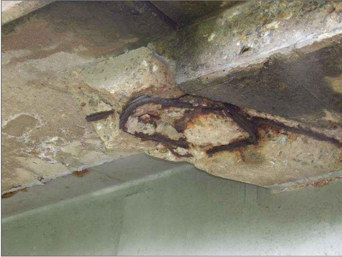
TYPICAL OVERHANG DIAPHRAGM SPALL 1 FEET LONG X 2 FEET WIDE X UP TO 4 INCH DEEP WITH EXPOSED REBAR WITH NO MEASURABLE SECTION LOSS, AT BENT 2 SHOWN
