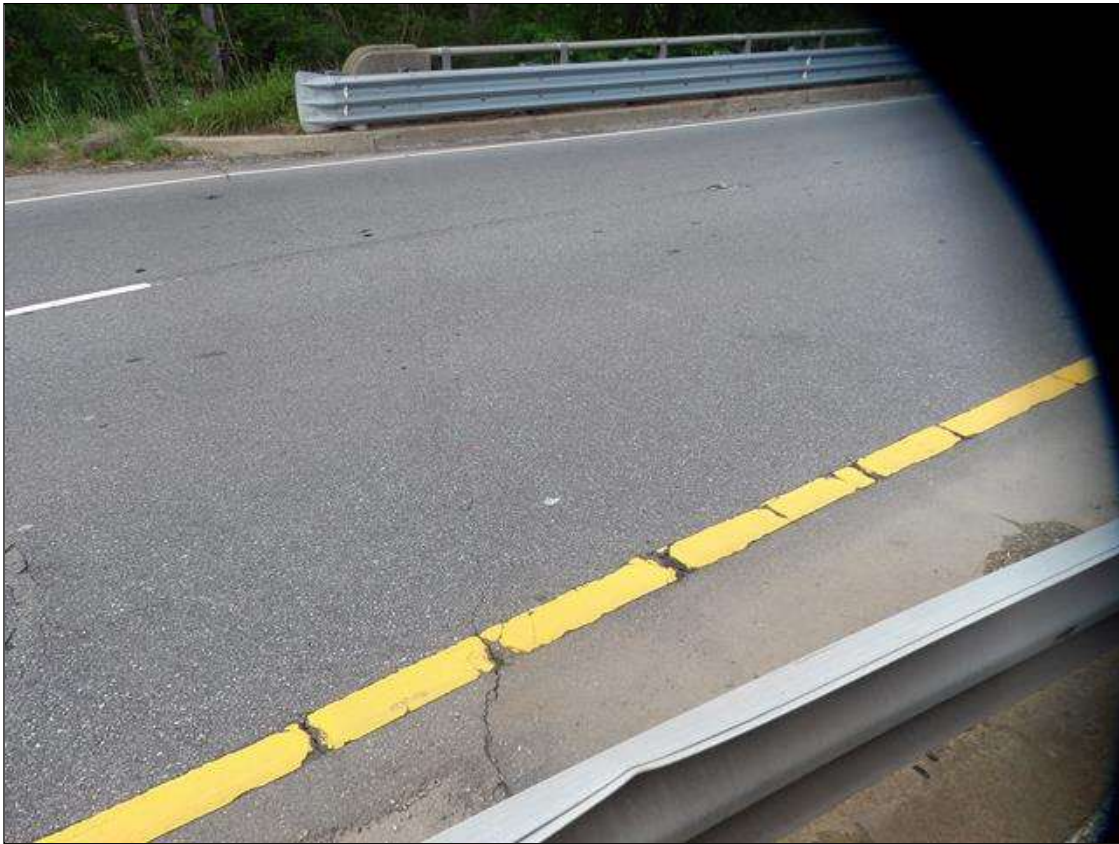
Span 1 Wearing Surface: UP TO 1/32 INCHES DIAGONAL CRACKS ALONG END BENT 1 FILL FACE IN INSIDE LANE
