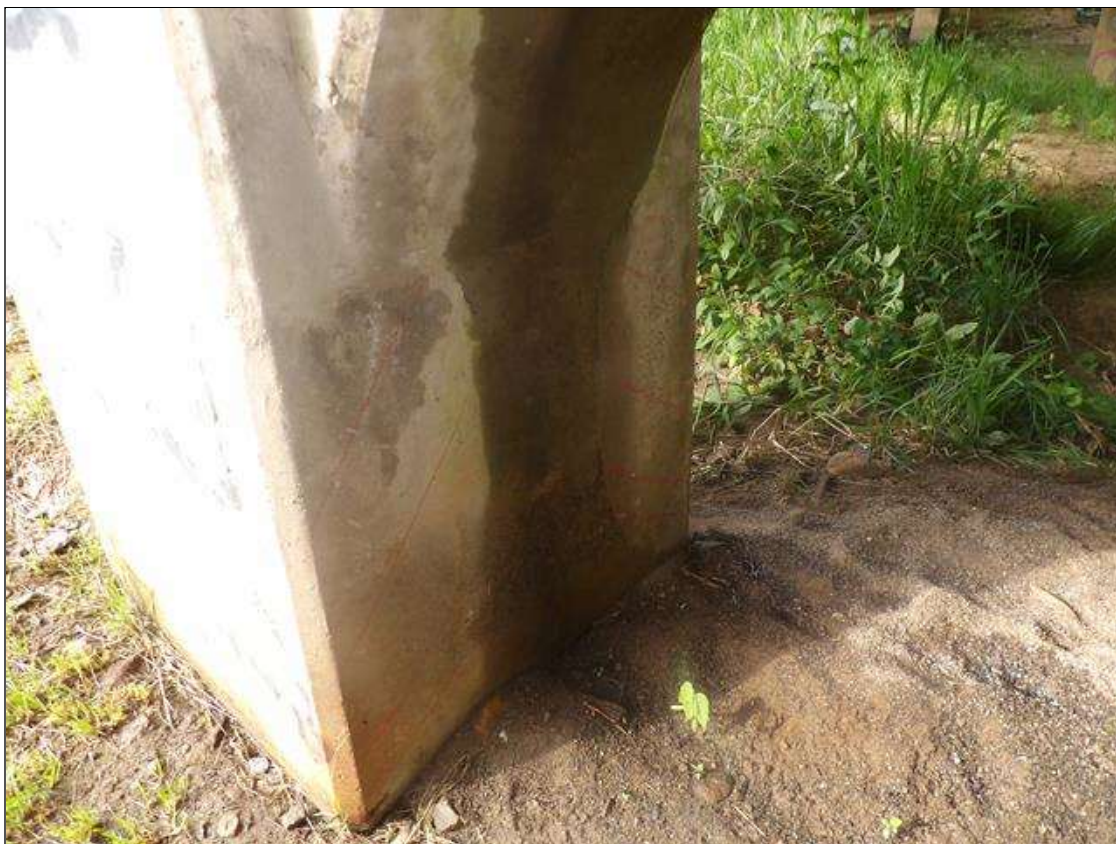
Bent 3 Pile 2: (2) AREAS OF DELAMINATION UP TO 33 INCHES X 9 INCHES X 9 INCHES WITH UP TO 1/16 INCHES VERTICAL CRACKS IN SOUTHWEST AND NORTHWEST CORNERS, APPROXIMATELY 3 FEET FROM BOTTOM OF CAP
