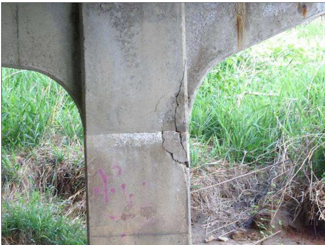
Bent 2 Pile 2: 40 INCHES X 9 INCHES X 6 INCHES AREA OF DELAMINATION WITH UP TO 3/8 INCHES VERTICAL CRACKS IN SOUTHEAST CORNER OF COLUMN, APPROXIMATELY 3 FEET FROM BOTTOM OF CAP
