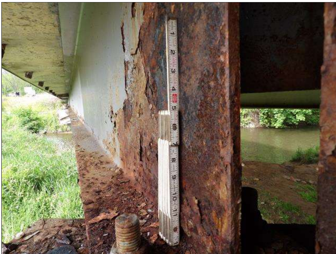
Span 3 Beam 4: 2 FOOT LONG CORROSION IN BOTTOM FLANG AND WEB WITH 1/16 INCH SECTION LOSS IN BOTTOM FLANGE FULL WIDTH WITH 9/16 INCH AVERAGE REMAINING AND UP TO 22 INCHES HIGH IN WEB WITH 1/16 INCH SECTION LOSS WITH 9/16 INCH AVERAGE REMAINING AT BENT 3
