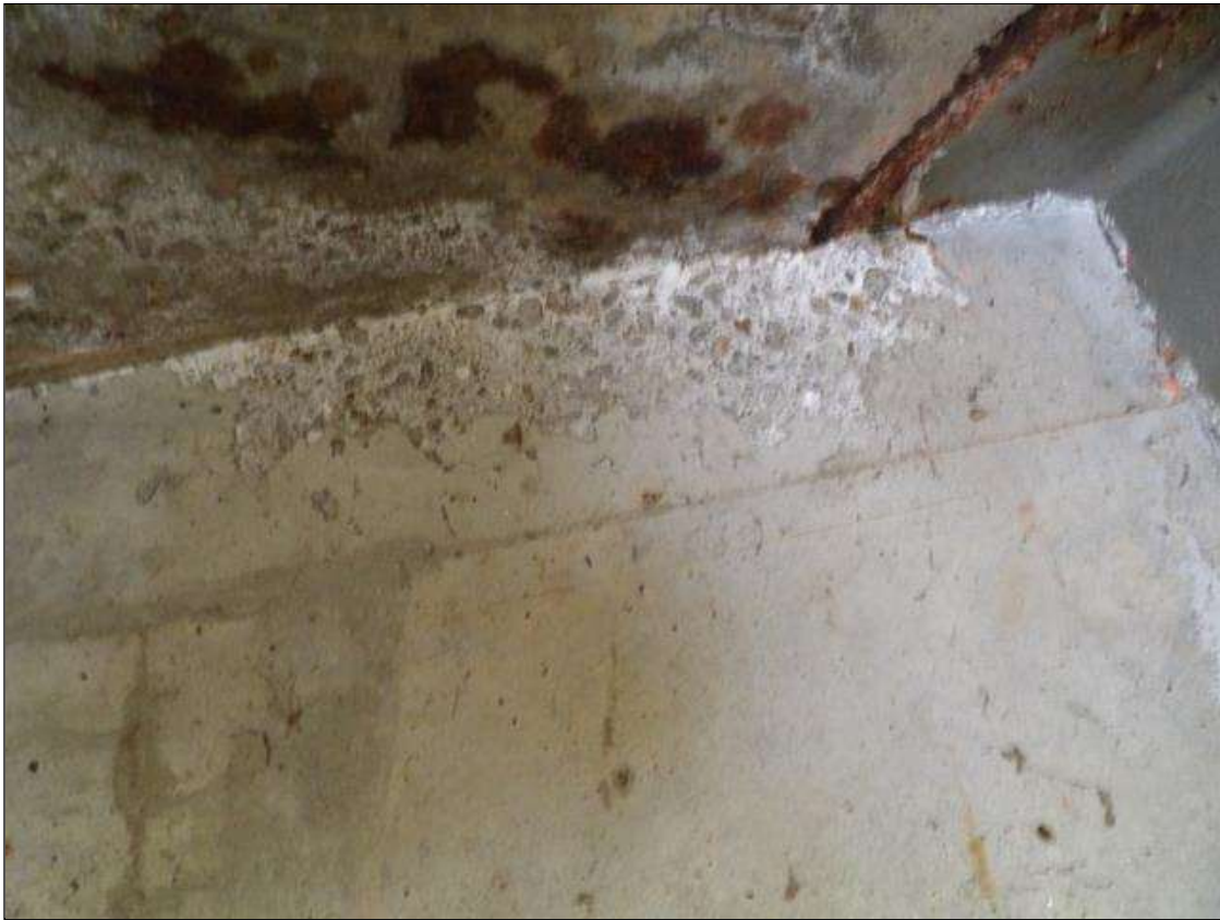
End Bent 1 Abutment: BELOW BAY 1 ADJACENT TO BEAM 1, 1 FOOT LONG X 4 INCHES HIGH X UP TO 1/4 INCHES DEEP SPALL
