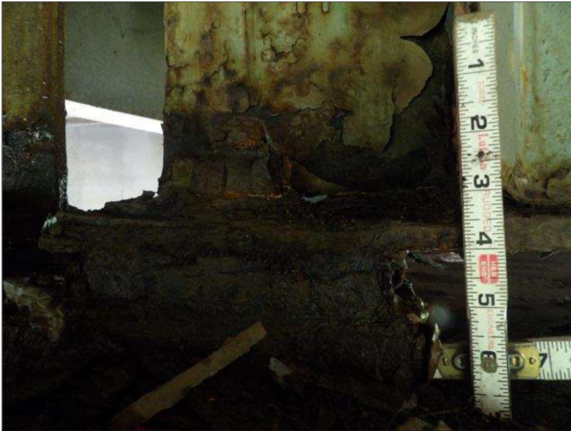
Span 3 Beam 2: CORROSION WITH 1/16 INCH SECTION LOSS ALONG LEFT EDGE OF BOTTOM FLANGE 9 INCHES LONG X 5 1/2 INCHES WIDE (9/16 INCH REMAINING) AT BENT 3
