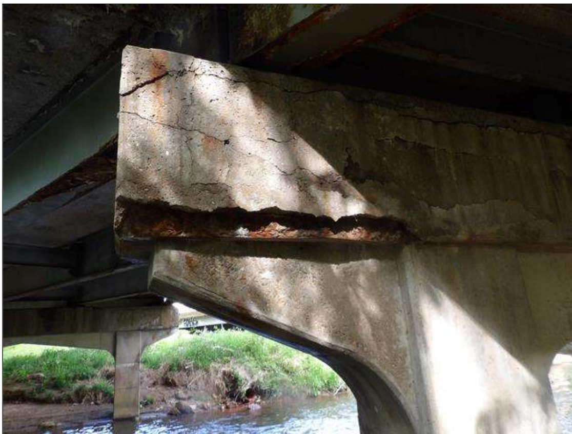
Bent 1 Cap 1: PAR: 50 INCHES X 4 INCHES X 5 INCHES SPALL WITH EXPOSED REBAR WITH MINOR SECTION LOSS IN BOTTOM AND SPAN 1 FACE OF CAP AT LEFT END
