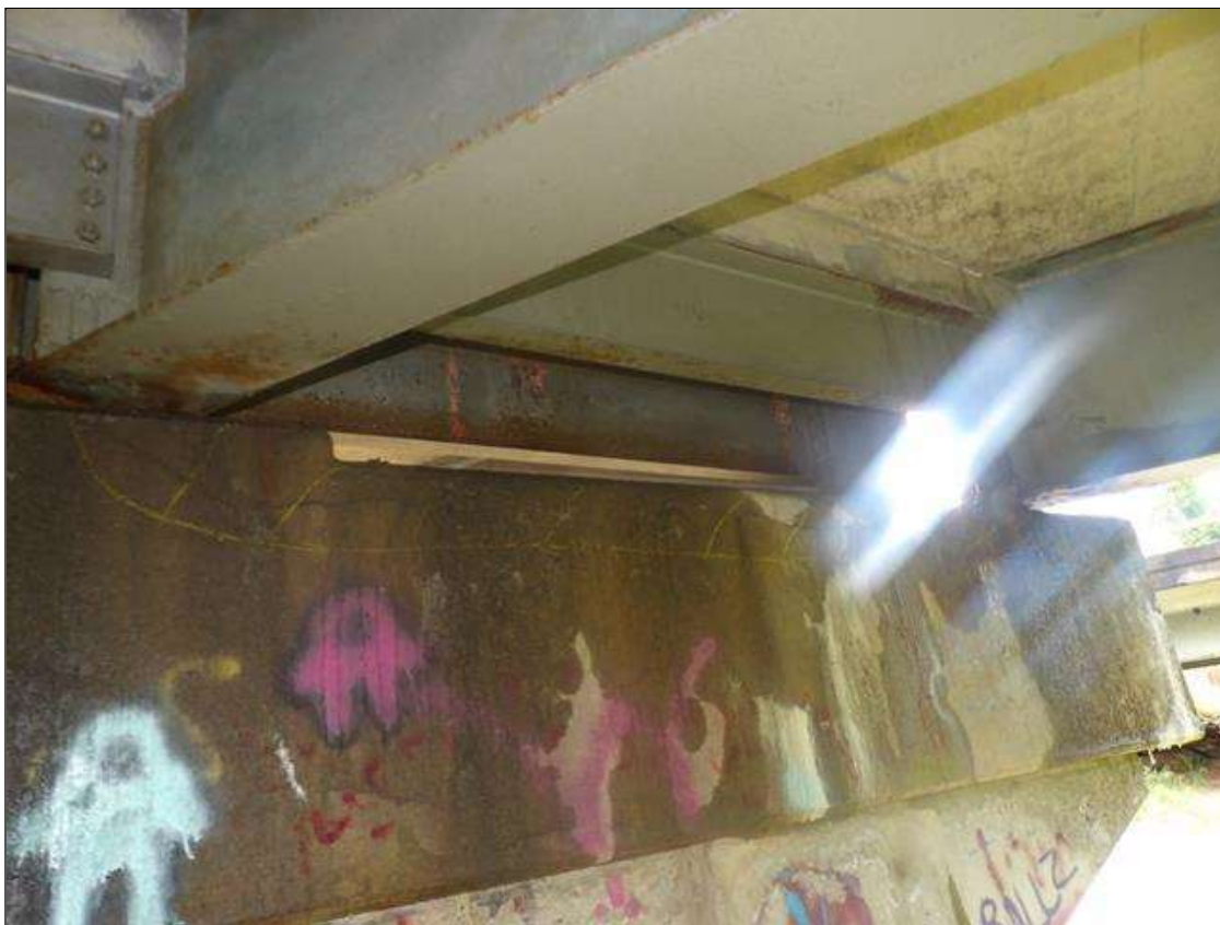
Bent 3 Cap 1: 7 FEET X 6 INCHES X 22 INCHES AREA OF DELAMINATION WITH UP TO 1/16 INCHES LONGITUDINAL AND HORIZONTAL CRACKS WITH AND WITHOUT EFFLORESCENCE IN TOP AND SPAN 3 FACE OF CAP BENEATH BAY 3
