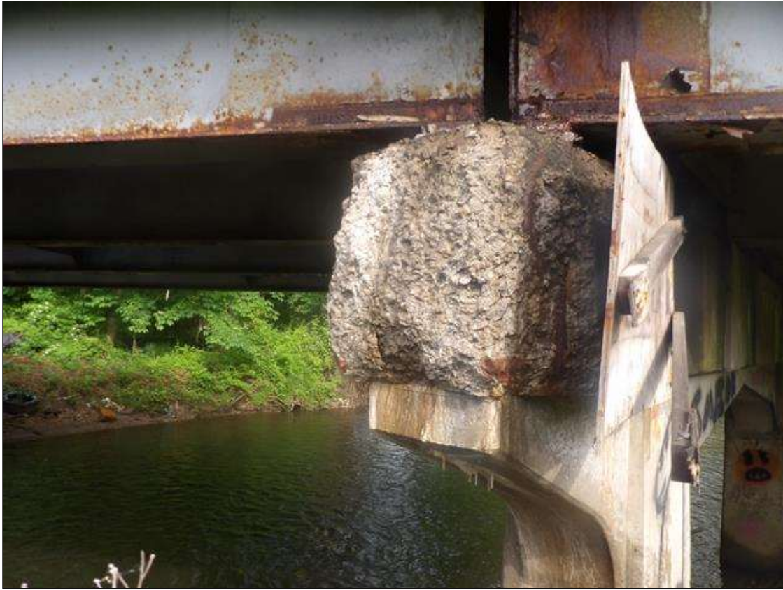
Bent 2 Cap 1: PAR: 30 INCHES X 30 INCHES X 12 INCHES DEEP SPALL WITH EXPOSED REBAR WITH MINOR SECTION LOSS AND FAILED REPAIR WITH 4 FEET SECTION OF FORMWORK IN RIGHT END OF CAP
