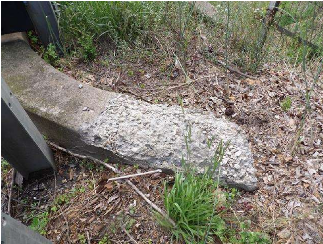
Span 4 Left Bridge Rail: END BENT 2 WHEEL GUARD EXTENSION, SPALL 3 FEET LONG X UP TO 12 INCHES WIDE X 2 INCHRS DEEP, RIGHT SIDE SIMILAR
