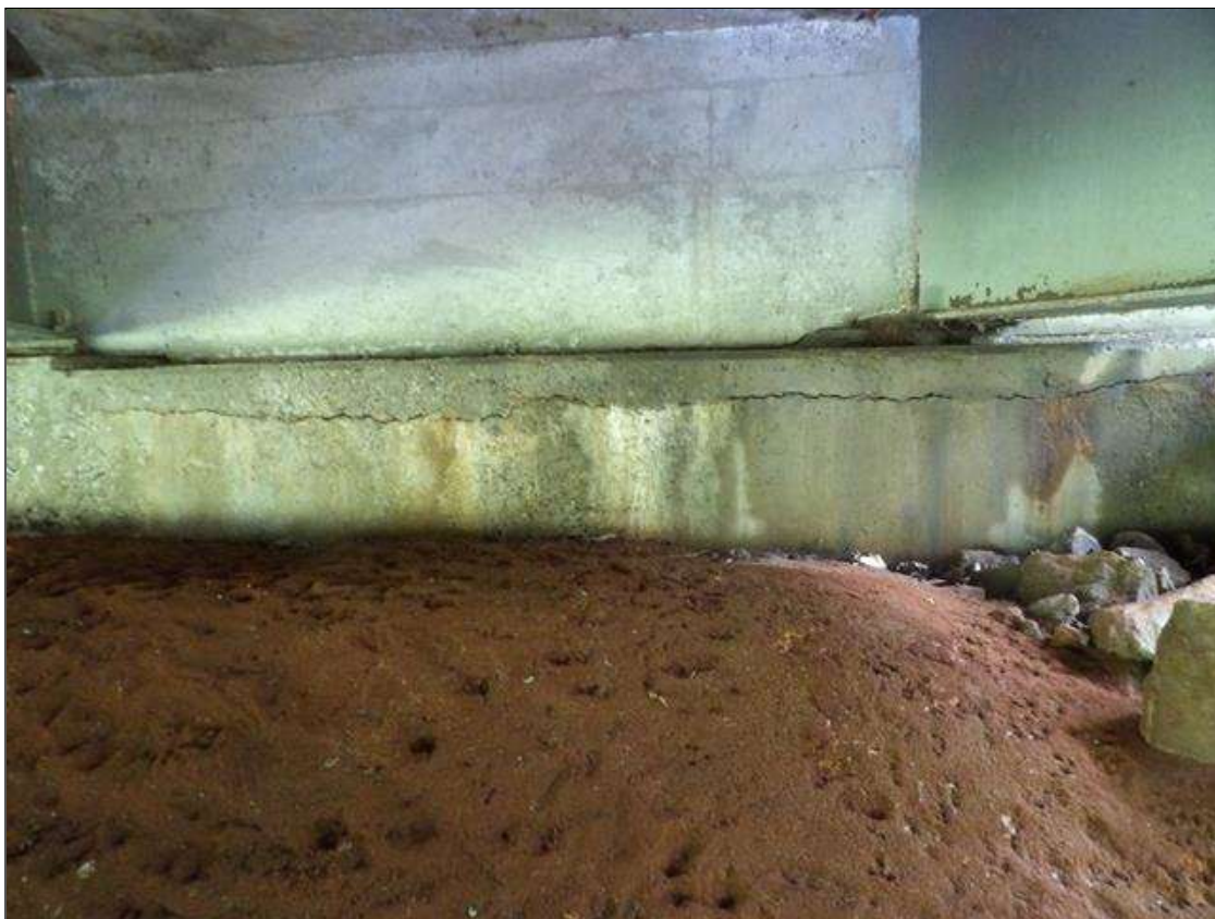
End Bent 1 Cap 1: 11 FEET X 18 INCHES X 8 INCHES AREA OF DELAMINATION WITH UP TO 3/8 INCHES HORIZONTAL CRACKS WITH AND WITHOUT EFFLORESCENCE IN TOP AND FACE OF CAP BENEATH BAY 1
