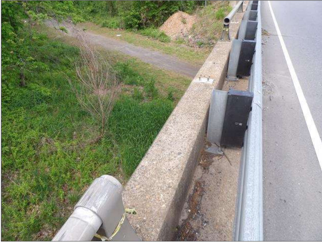
Span 3 Left Bridge Rail: 30 FEET SECTION OF IMPACT DAMAGE WITH SEPARATED, CRACKED AND MISSING RAIL AND RAIL POSTS EXTENDING FROM BENT 3; CONDITION MITIGATED WITH ADDITION OF THREE BEAM METAL RAIL
