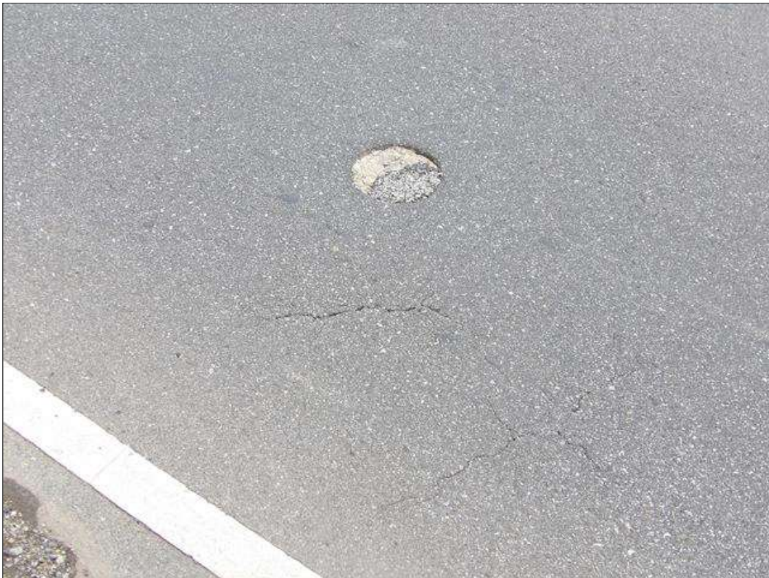
Span 1 Wearing Surface: 8 INCHES DIAMETER PATCHED CORED HOLE IN OUTSIDE LANE, APPROXIMATELY 15 FEET FROM BENT 1
