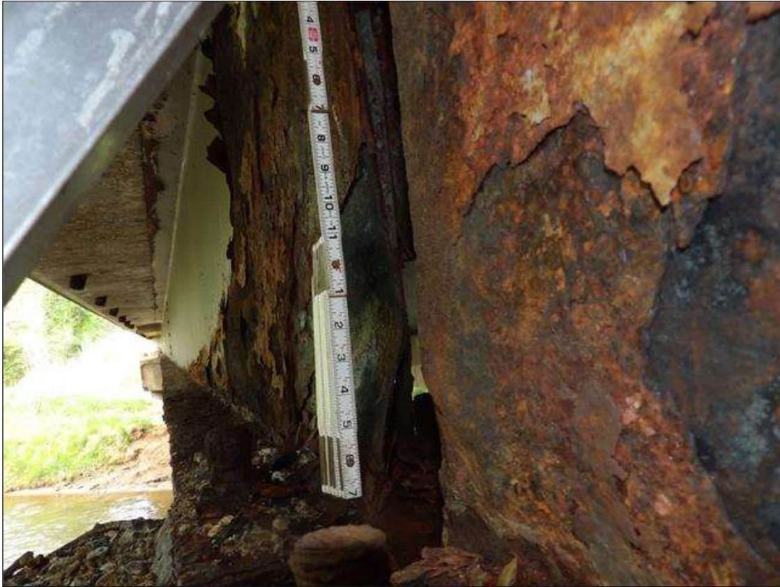
Span 2 Beam 1: PAR: CORROSION ALONG BOTH FACES OF WEB AND BOTTOM FLANGE. WEB: UP TO 8 FEET LONG X FULL HEIGHT DOWN TO 1/8 INCHES RESIDUAL WEB WITH 4 INCHES WIDE X 7 INCHES HIGH X 1/2 INCHES DEEP BUCKLING AT THE BASE OF THE WEB. 8 FEET LONG X FULL WIDTH DOWN TO 1/16 INCHES RESIDUAL FLANGE AT BENT 1.
