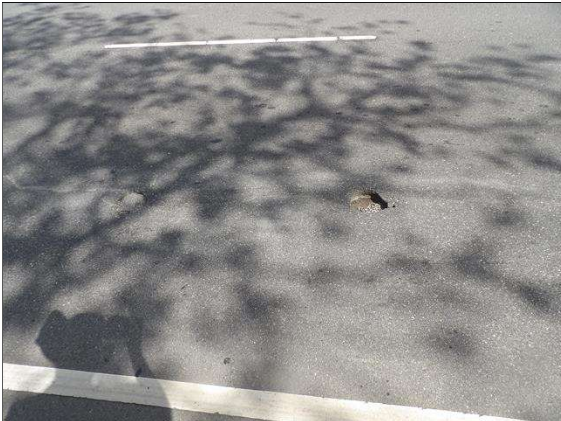
NORTH APPROACH ROADWAY WITH TWO 8 INCH DIAMETER CORES WITH ASPHALT MISSING UP TO 6 INCHES DEEP, SOUTH APPROACH SIMILAR
