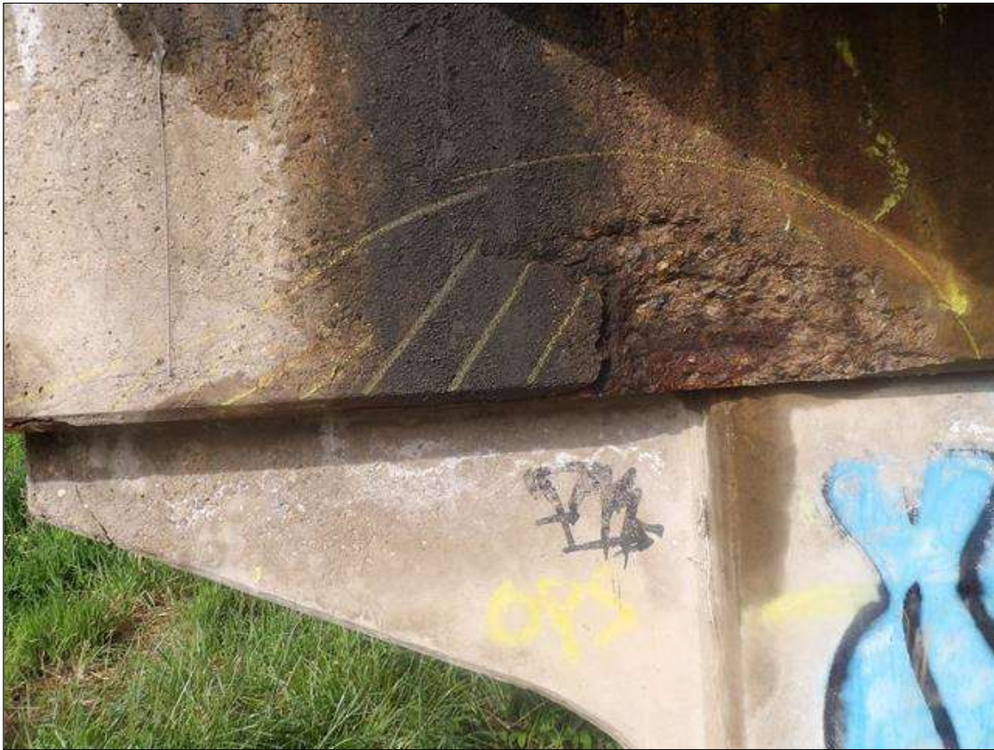
Bent 3 Cap 1: PAR: 26 INCHES X 2 INCHES X 11 INCHES SPALL WITH EXPOSED REBAR WITH MINOR SECTION LOSS AND 45 INCHES X 9 INCHES X 6 INCHES AREA OF DELAMINATION WITH UP TO 1/4 INCHES LONGITUDINAL AND HORIZONTAL CRACKS IN BOTTOM AND SPAN 4 FACE OF CAP AT RIGHT END
