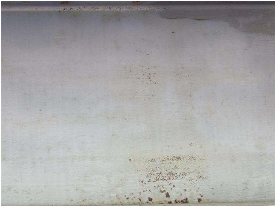
TYPICAL AREAS OF SURFACE CORROSION THROUGHOUT BEAM, SPAN 4 BEAM 3 SHOWN
