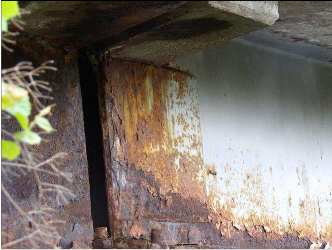
BEAM 4 SPAN 2 WITH WELDED PLATE REPAIRS ON RIGHT FACE OF WEB AND BOTTOM FLANGE 24 INCHES LONG X 24 INCHES HIGH X 1/2 INCH THICK IN WEB, AND 24 INCHES LONG X 4 INCHES X 1/2 INCH WIDE IN FLANGE AT BENT 1
