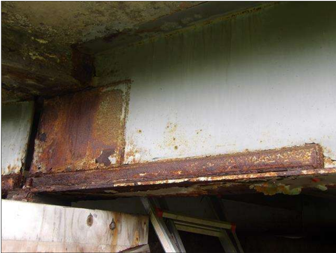
SPAN 3 BEAM 4 AT BENT 2 WELDED PLATE REPAIRS ON BOTH FACES OF WEB AND BOTTOM FLANGE UP TO 60 INCHES LONG X 21 1/2 INCHES HIGH X 1/2 INCH THICK IN WEB, AND 60 INCHES LONG X 4 INCHES WIDE X 1/2 INCH THICK IN FLANGE AT BENT 2
