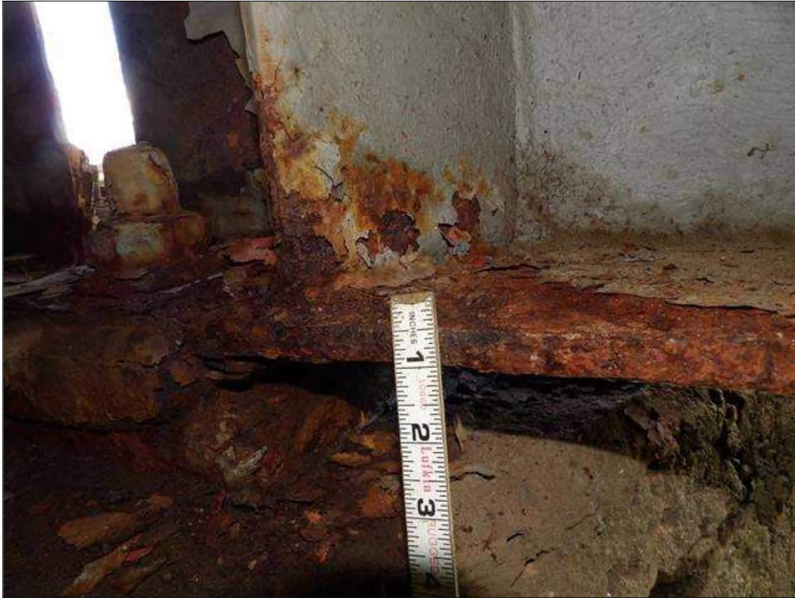
Span 1 Beam 4: PAR: CORROSION ALONG BOTH FACES OF WEB AND BOTTOM FLANGE UP TO 60 INCHES LONG X 31 1/2 INCHES HIGH DOWN TO 7/16 INCHES RESIDUAL WEB, AND 60 INCHES LONG X 11 5/8 INCHES WIDE DOWN TO 5/16 INCHES RESIDUAL FLANGE AT BENT 1
