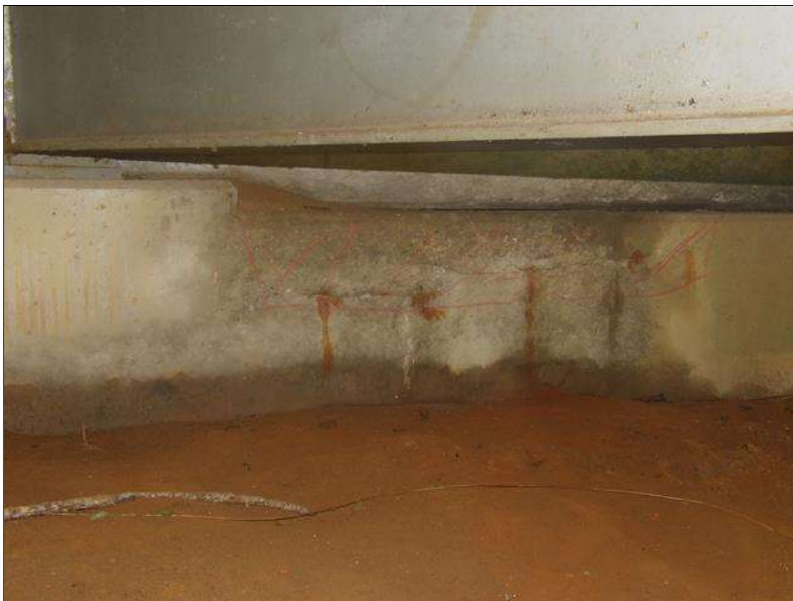
End Bent 2 Cap 1: 46 INCHES X 8 INCHES X 9 INCHES AREA OF DELAMINATION WITH UP TO 1/16 INCHES LONGITUDINAL AND HORIZONTAL CRACKS WITH AND WITHOUT EFFLORESCENCE IN TOP AND FACE OF CAP BENEATH BAY 3
