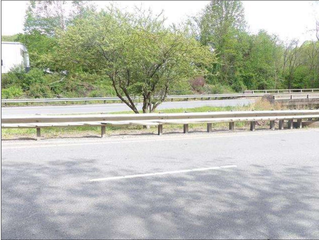
NORTHEAST GUARDRAIL IMPACT DAMAGE 50 FOOT LONG WITH TEARS IN GUARDRAIL STARTING AT ABUTMENT 2
