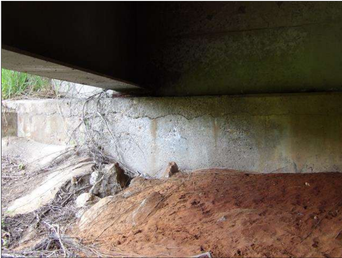
End Bent 1 Cap 1: UP TO 3/8 INCHES HORIZONTAL CRACK WITH AND WITHOUT EFFLORESCENCE AND 86 INCHES X 14 INCHES X 8 INCHES AREA OF DELAMINATION IN TOP AND FACE OF CAP BENEATH BAY 3 AND BEAM 4
