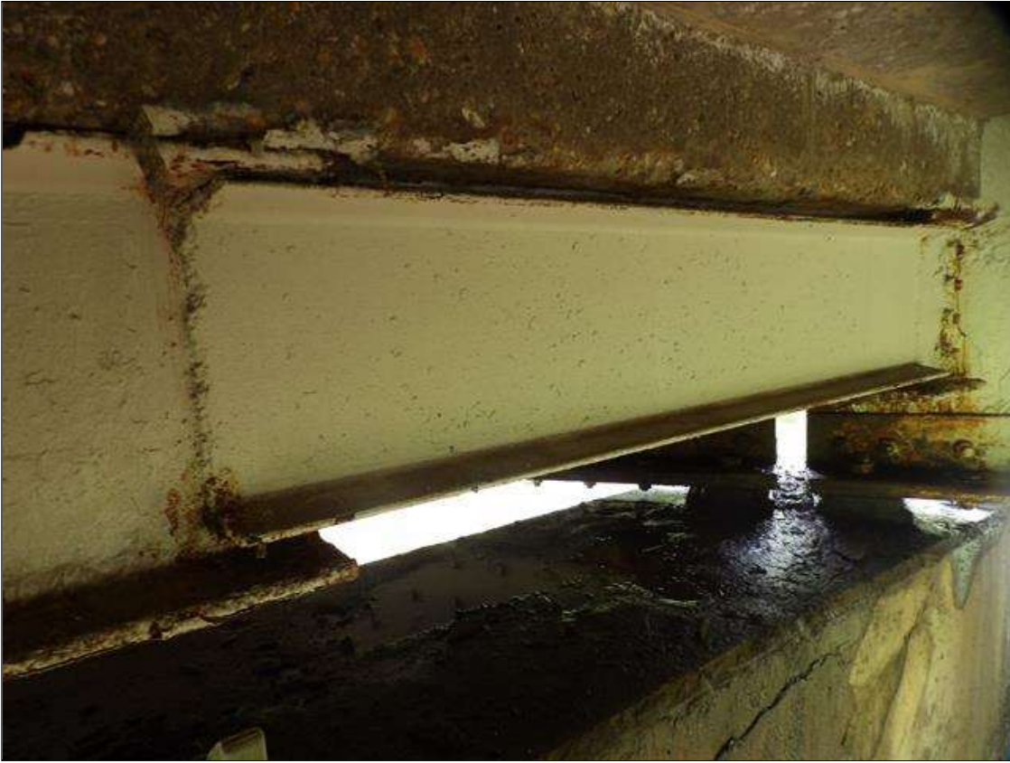
SPAN 3 BENT 2 DIAPHRAGM IN BAY 1, 5 FEET LONG SECTION HAS BEEN REPLACED WITH 12 INCHES X 3 INCHES STEEL CHANNEL WELDED AT EACH END
