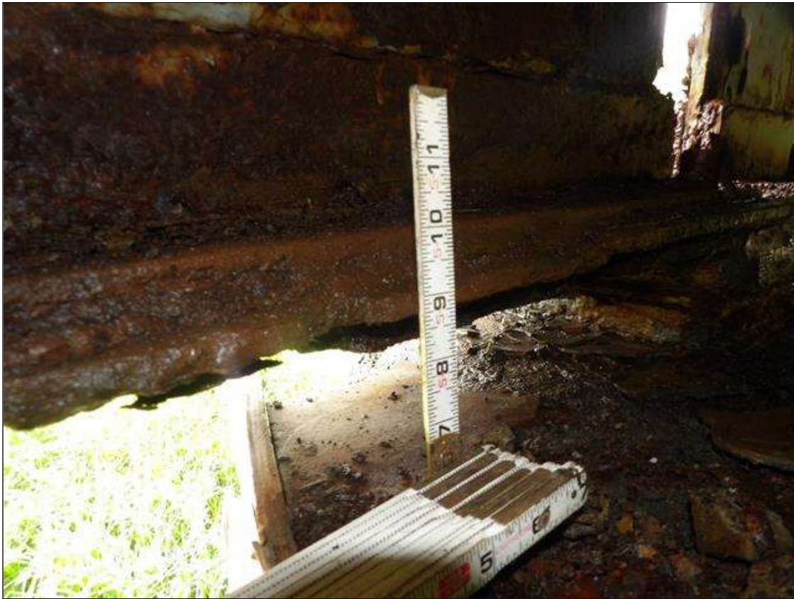
Span 3 Beam 4: PAR--6 FOOT LONG CORROSION IN BOTTOM FLANGE REPAIR PLATE WITH 1/4 INCH AVERAGE REMAINING WITH 1 1/2 INCH X 1/2 INCH HOLE IN LEFT SIDE AT 18 INCHES FROM BEARING, BOTTOM FLANGE BELOW REPAIR PLATE WITH 3/8 INCH AVERAGE REMAINING WITH 24 INCH X UP TO 1 1/2 INCH WIDE HOLE IN LEFT SIDE STARTING AT BEARING. MEASUREMENTS OF WELDED PLATE REPAIRS ON BOTH FACES OF WEB AND BOTTOM FLANGE UP TO 60 INCHES LONG X 21 1/2 INCHES HIGH X 1/2 INCH THICK IN WEB, AND 60 INCHES LONG X 4 INCHES WIDE X 1/2 INCH THICK IN FLANGE AT BENT 2
