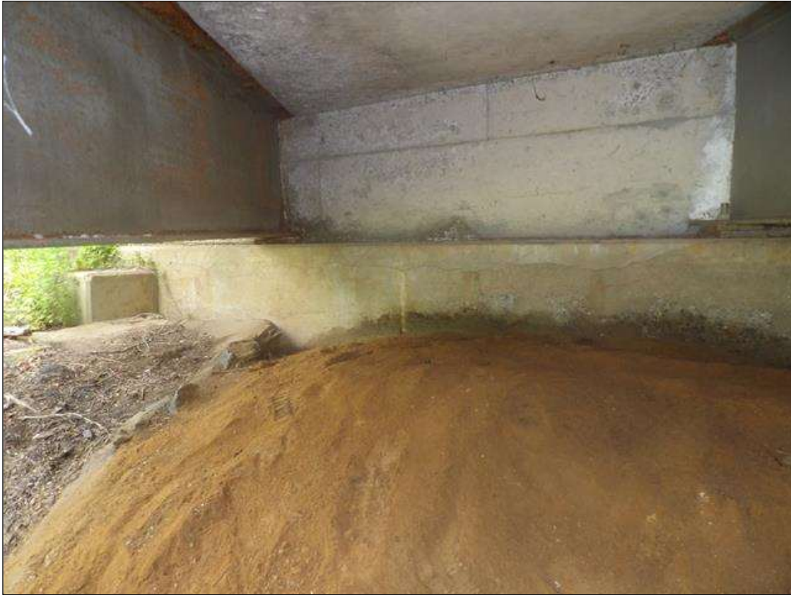
End Bent 2 Cap 1: 13 FEET X 15 INCHES X 8 INCHES AREA OF DELAMINATION WITH UP TO 1/16 INCHES LONGITUDINAL AND HORIZONTAL CRACKS WITH AND WITHOUT EFFLORESCENCE IN TOP AND FACE OF CAP FROM LEFT OF BEAM 1 TO BEAM 2
