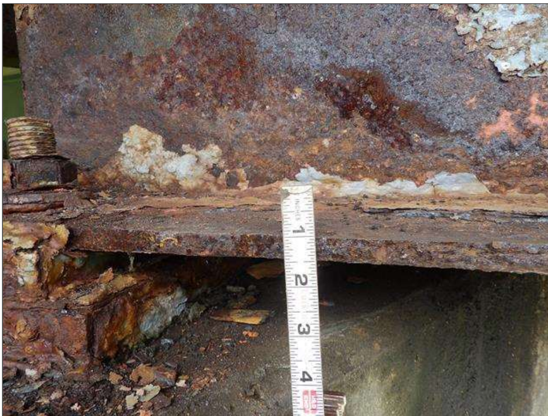
Span 4 Beam 4: CORROSION ALONG BOTH FACES OF WEB AND BOTTOM FLANGE UP TO 36 INCHES LONG X 13 INCHES HIGH WITH NO MEASURABLE LOSS OF SECTION IN WEB, AND 36 INCHES LONG X 5 1/2 INCHES WIDE DOWN TO 7/16 INCHES RESIDUAL WITH 1/2 INCH AVERAGE REMAINING IN FLANGE AT BENT 3
