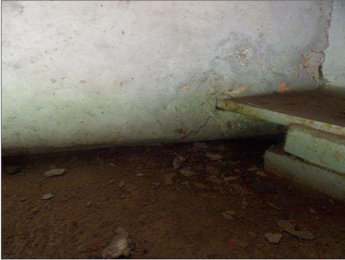
End Bent 2 Abutment: UP TO 1/16 INCHES DIAGONAL CRACKS IN FACE OF CURTAIN WALL EXTENDING FROM LEFT EDGE OF BOTTOM FLANGE OF BEAMS 1, 3 AND 4
