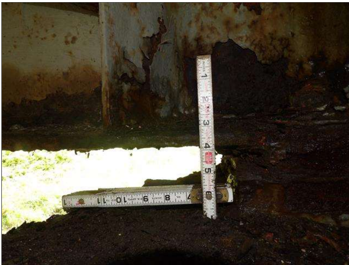
Span 4 Beam 2: CORROSION WITH 1/16 INCH SECTION LOSS ALONG LEFT EDGE OF BOTTOM FLANGE 20 INCHES LONG X 11 5/8 INCHES WIDE (9/16 INCH REMAINING) AND CORROSION WITH NO MEASURABLE LOSS OF SECTION ALONG BOTH FACES OF WEB UP TO 27 INCHES LONG X 5 INCHES HIGH IN WEB AT BENT
