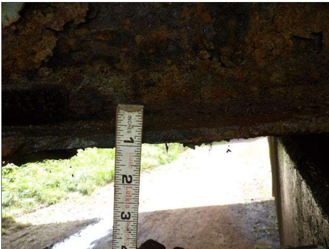
Span 4 Beam 1: PAR: CORROSION ALONG BOTH FACES OF WEB AND BOTTOM FLANGE UP TO 72 INCHES LONG X 31 1/2 INCHES HIGH DOWN TO 7/16 INCHES RESIDUAL WEB, AND 82 INCHES LONG X 11 5/8 INCHES WIDE DOWN TO 3/8 INCHES RESIDUAL FLANGE AT BENT 3
