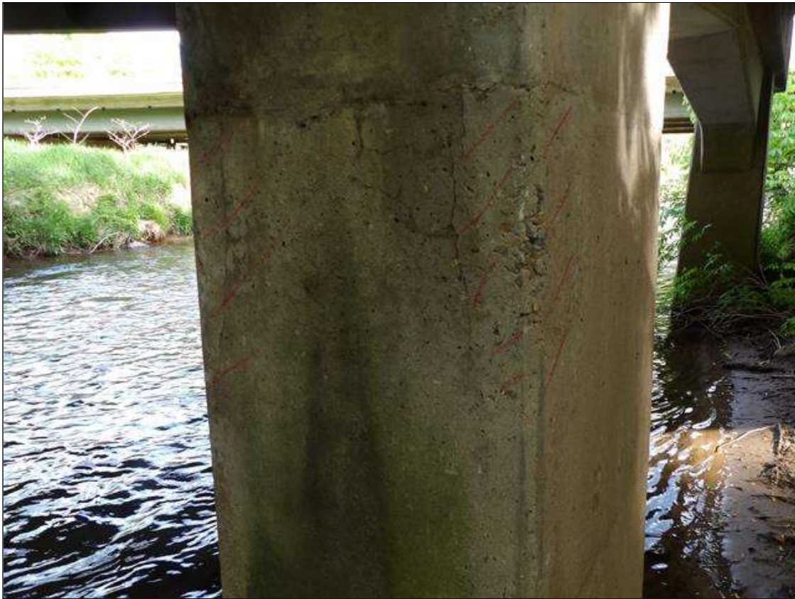
Bent 1 Pile 1: (2) AREAS OF DELAMINATION UP TO 24 INCHES X 5 INCHES X 5 INCHES WITH 1/32 INCHES VERTICAL CRACKS IN SOUTHWEST AND NORTHWEST CORNERS OF COLUMN, APPROXIMATELY 3 FEET FROM BOTTOM OF CAP
