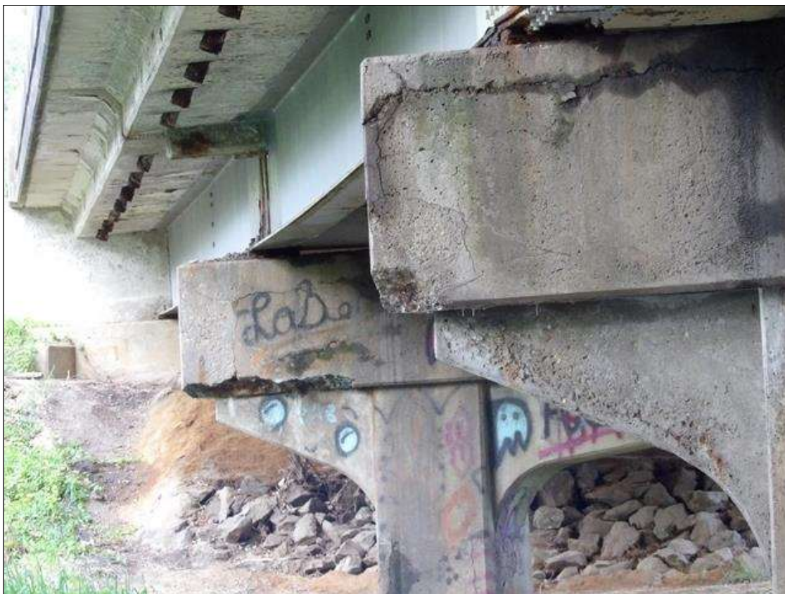
Bent 2 Cap 1: LEFT END OF CAP, DELAMINATED AREA FULL HEIGHT AND FULL WIDTH WITH CRACKING UP 1/4 INCH WITH 8 INCH DIAMETER X 2 INCH DEEP SPALL AT SOUTHWEST CORNER
