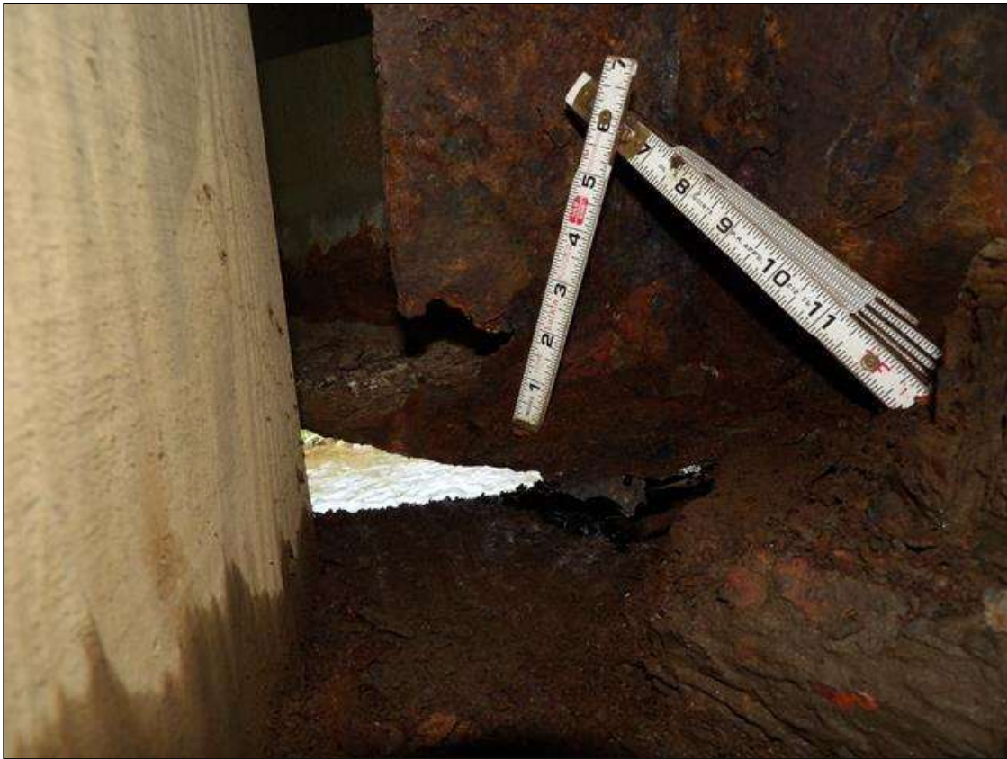
Span 2 Beam 4: PAR: CORROSION ALONG BOTH FACES OF WEB, BOTTOM FLANGE AND LEFT STIFFENER UP TO 60 INCHES LONG X 31 1/2 INCHES HIGH DOWN TO 1/2 INCHES RESIDUAL WEB, 66 INCHES LONG X 11 5/8 INCHES WIDE DOWN TO KNIFE'S EDGE RESIDUAL FLANGE WITH 2 INCHES X 3 INCHES LOSS OF SECTION, AND 10 INCHES HIGH X 5 INCHES WIDE DOWN TO KNIFE'S EDGE RESIDUAL STIFFENER WITH 1 INCHES DIAMETER HOLE AT BENT 1; TIMBER BLOCK ADDED ADJACENT TO BEAM
