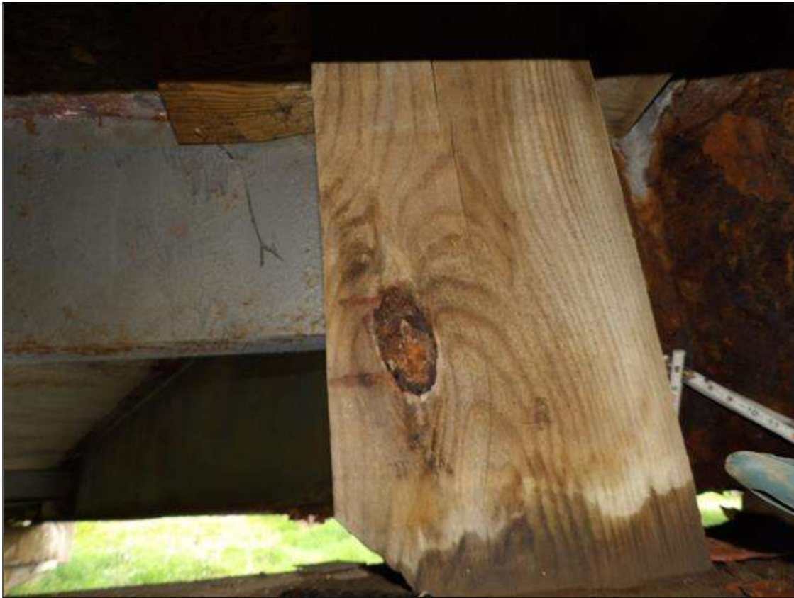
Span 2 Beam 4: PAR: CORROSION ALONG BOTH FACES OF WEB, BOTTOM FLANGE AND LEFT STIFFENER UP TO 60 INCHES LONG X 31 1/2 INCHES HIGH DOWN TO 1/2 INCHES RESIDUAL WEB, 66 INCHES LONG X 11 5/8 INCHES WIDE DOWN TO KNIFE'S EDGE RESIDUAL FLANGE WITH 2 INCHES X 3 INCHES LOSS OF SECTION, AND 10 INCHES HIGH X 5 INCHES WIDE DOWN TO KNIFE'S EDGE RESIDUAL STIFFENER WITH 1 INCHES DIAMETER HOLE AT BENT 1; TIMBER BLOCK ADDED ADJACENT TO BEAM
