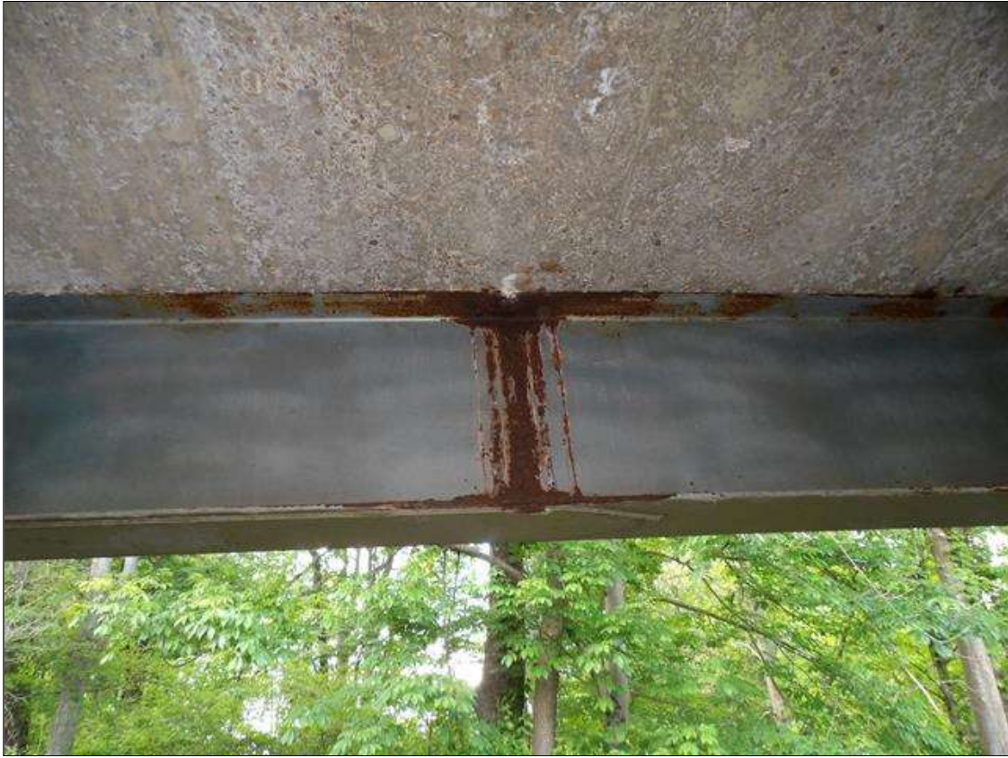
TYPICAL AREAS OF SURFACE CORROSION AND CORROSION WITH NO MEASURABLE SECTION LOSS THROUGHOUT BEAM, BEAM 1 SPAN 1 SHOWN
