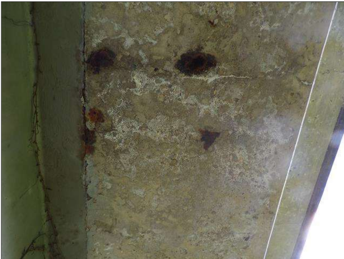
Span 1 Deck: ALONG BOTH OVERHANG DECK SOFFITS, HAIRLINE MAP CRACKING WITH ABRASION UP TO 1/16 INCH DEEP WITH EXPOSED BUT SECURE AGGREGATE AND EFFLORESCENCE AND RUST STAINING
