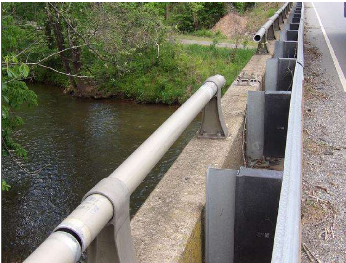
Span 1 Left Bridge Rail: 10 FEET SECTION OF IMPACT DAMAGE WITH MISSING RAIL AND RAIL POST EXTENDING FROM BENT 1; CONDITION MITIGATED WITH ADDITION OF THRIE BEAM METAL RAIL
