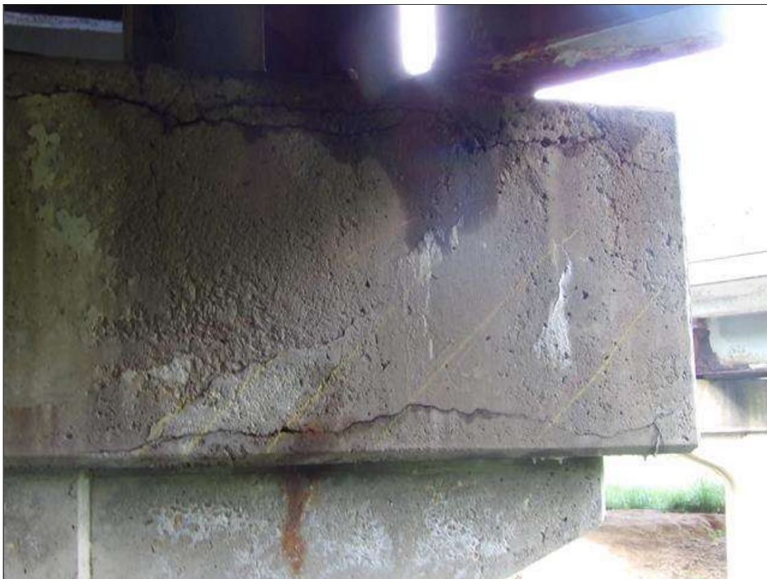
Bent 1 Cap 1: DELAMINATED AREA 30 INCHES WIDE X 14 INCHES HIGH ON SOUTH FACE NEAR RIGHT END.
