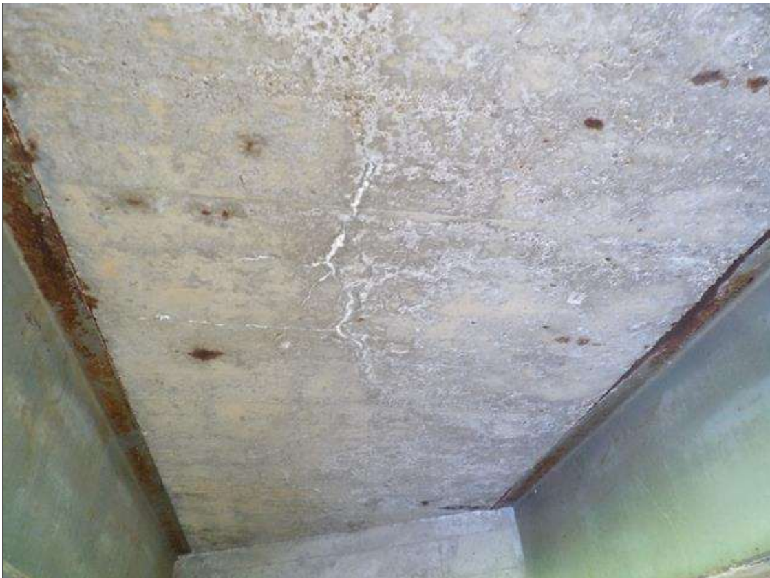
Span 1 Deck: UP TO 1/32 INCHES TRANSVERSE AND LONGITUDINAL AND HAIRLINE MAP CRACKS WITH AND WITHOUT EFFLORESCENCE IN BOTTOM OF DECK IN VARIOUS LOCATIONS
