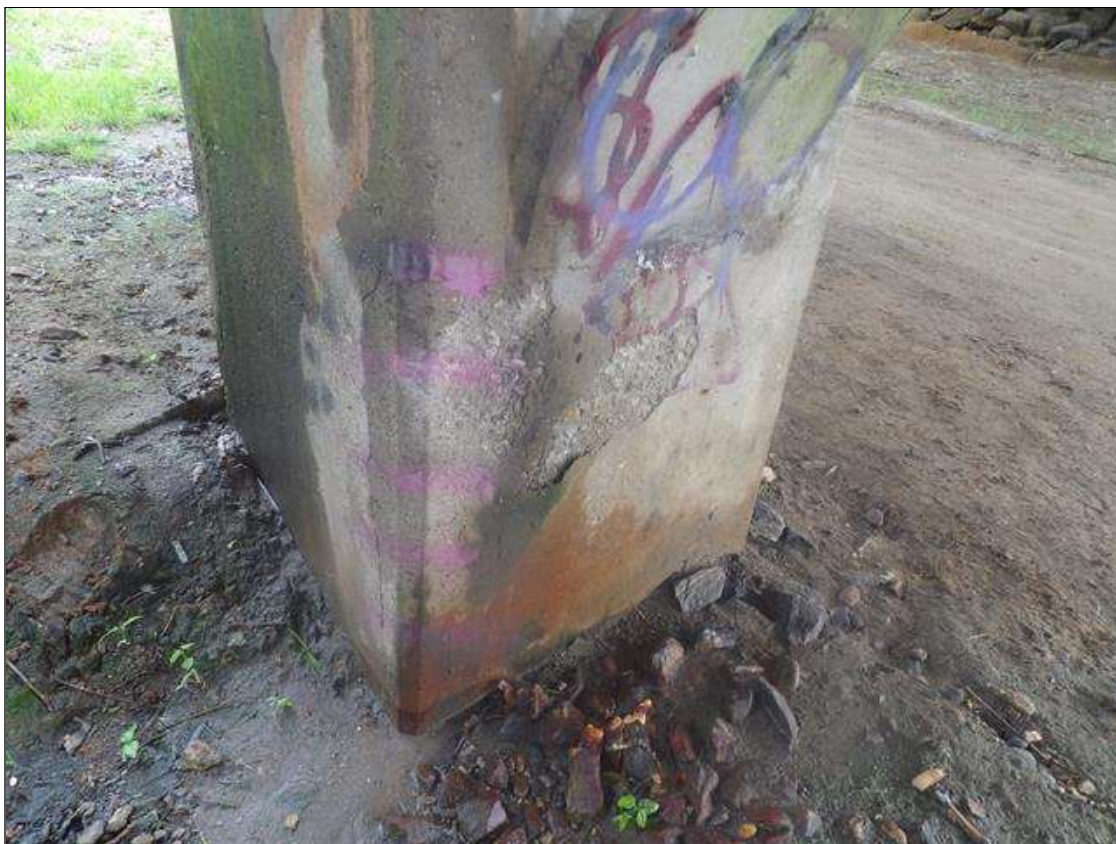
Bent 3 Pile 1: WEST FACE STARTING AT BOTTOM OF PILE, SPALL 2 FEET HIGH X 1 FEET WIDE X UP TO 1/8 INCH DEEP
