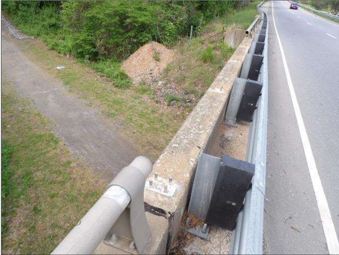
Span 4 Left Bridge Rail: 25 FEET SECTION OF IMPACT DAMAGE WITH MISSING RAIL AND RAIL POSTS EXTENDING FROM BENT 3; CONDITION MITIGATED WITH ADDITION OF THRIE BEAM METAL RAIL
