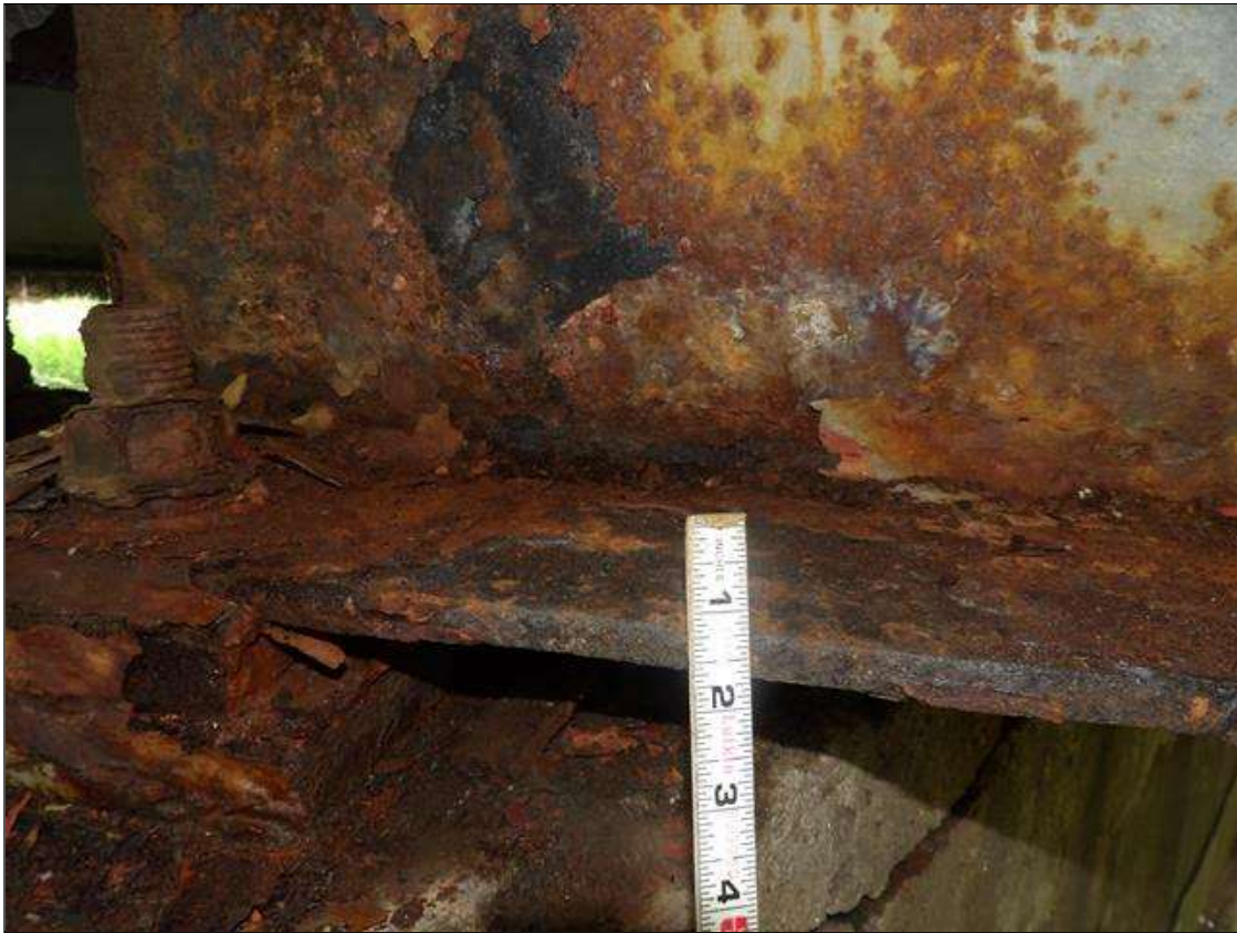
Span 1 Beam 1: PAR: CORROSION ALONG BOTTOM FLANGE AND WEB. FLANGE REDUCED TO 3/16 INCHES WITH 1/2 INCH AVERAGE REMAINING FOR 36 INCHES LONG X 11 5/8 INCHES WIDE BEGINNING AT FAR END. WEB ALSO REDUCED TO 3/8 INCHES WITH 7/16 INCH AVERAGE REMAINING THE FULL HEIGHT X 11 INCHES LONG BEGINNING AT THE FAR END.
