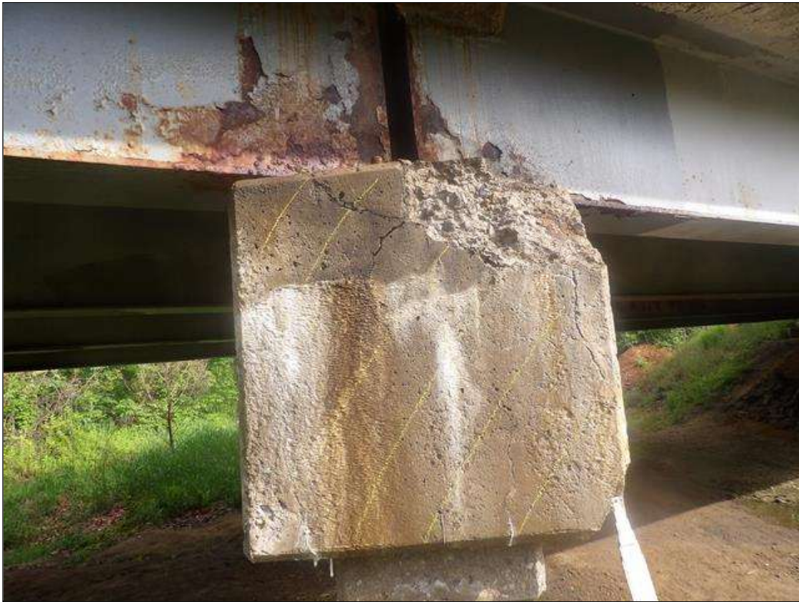
Bent 3 Cap 1: 32 INCHES X 30 INCHES X 30 INCHES AREA OF DELAMINATION WITH UP TO 1/4 INCHES HORIZONTAL AND MAP CRACKS AND 10 INCHES X 9 INCHES X 6 INCHES DEEP SPALL WITH EXPOSED REBAR NO LOSS THROUGHOUT RIGHT END OF CAP
