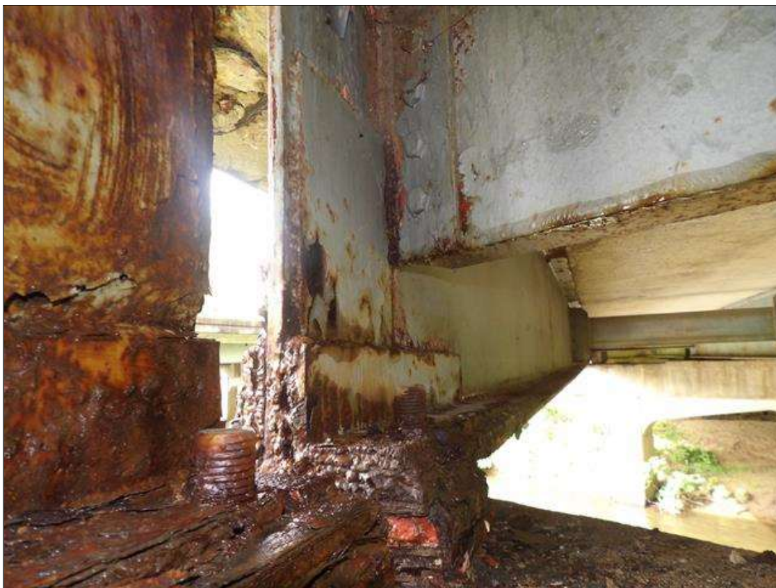
SPAN 2 BEAM 4 AT BENT 2 WELDED PLATE REPAIRS ON BOTH FACES OF WEB AND BOTTOM FLANGE UP TO 30 INCHES LONG X 14 INCHES HIGH X 1/2 INCH THICK IN WEB, AND 30 INCHES LONG X 4 INCHES WIDE X 1/2 INCH THICK IN FLANGE AT BENT 2
