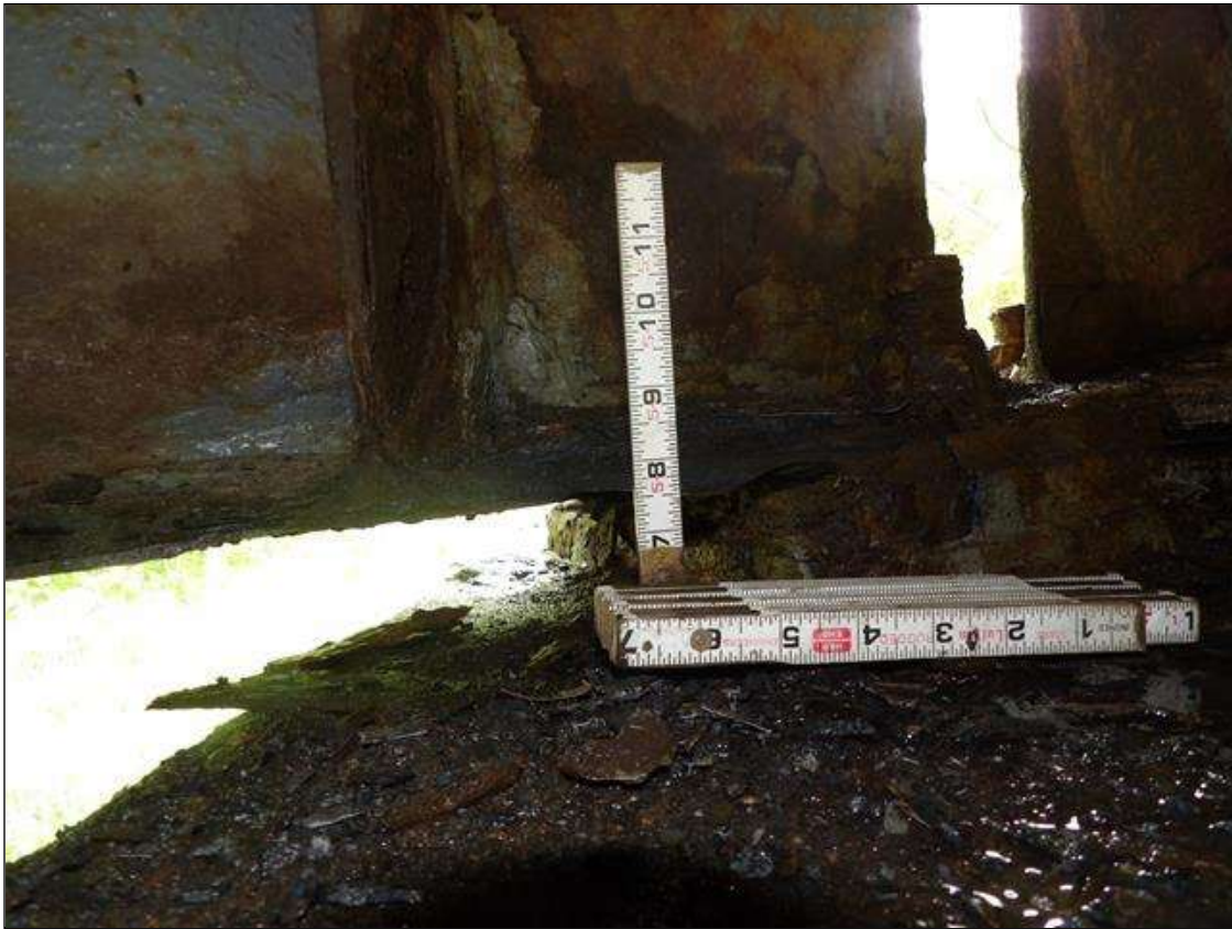
Span 3 Beam 1: PAR: CORROSION ALONG BOTH FACES OF WEB AND BOTTOM FLANGE UP TO 43 INCHES LONG X 10 INCHES HIGH DOWN TO 1/2 INCHES RESIDUAL WEB, AND 36 INCHES LONG X UP TO 11 INCHES WIDE WITH SECTION LOSS DOWN TO KNIFES EDGE WITH 1/4 INCH AVERAGE REMAINING FULL WIDTH OF FLANGE WITH 8 INCH X 2 INCH AREA AT BEARING THAT IS PAPER THIN WITH PERFORATIONS ON RIGHT SIDE AT BENT 3
