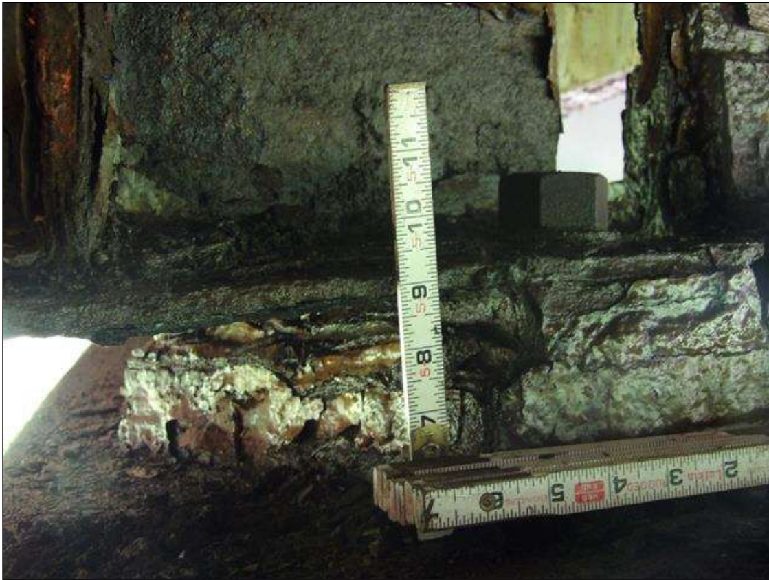
Span 3 Beam 2: PAR: CORROSION ALONG BOTH FACES OF WEB AND BOTTOM FLANGE UP TO 10 INCHES LONG X 4 INCHES HIGH DOWN TO 1/4 INCHES RESIDUAL WEB, AND 12 INCHES LONG X 5 1/2 INCHES WIDE DOWN TO 3/8 INCHES RESIDUAL FLANGE AT BENT 2
