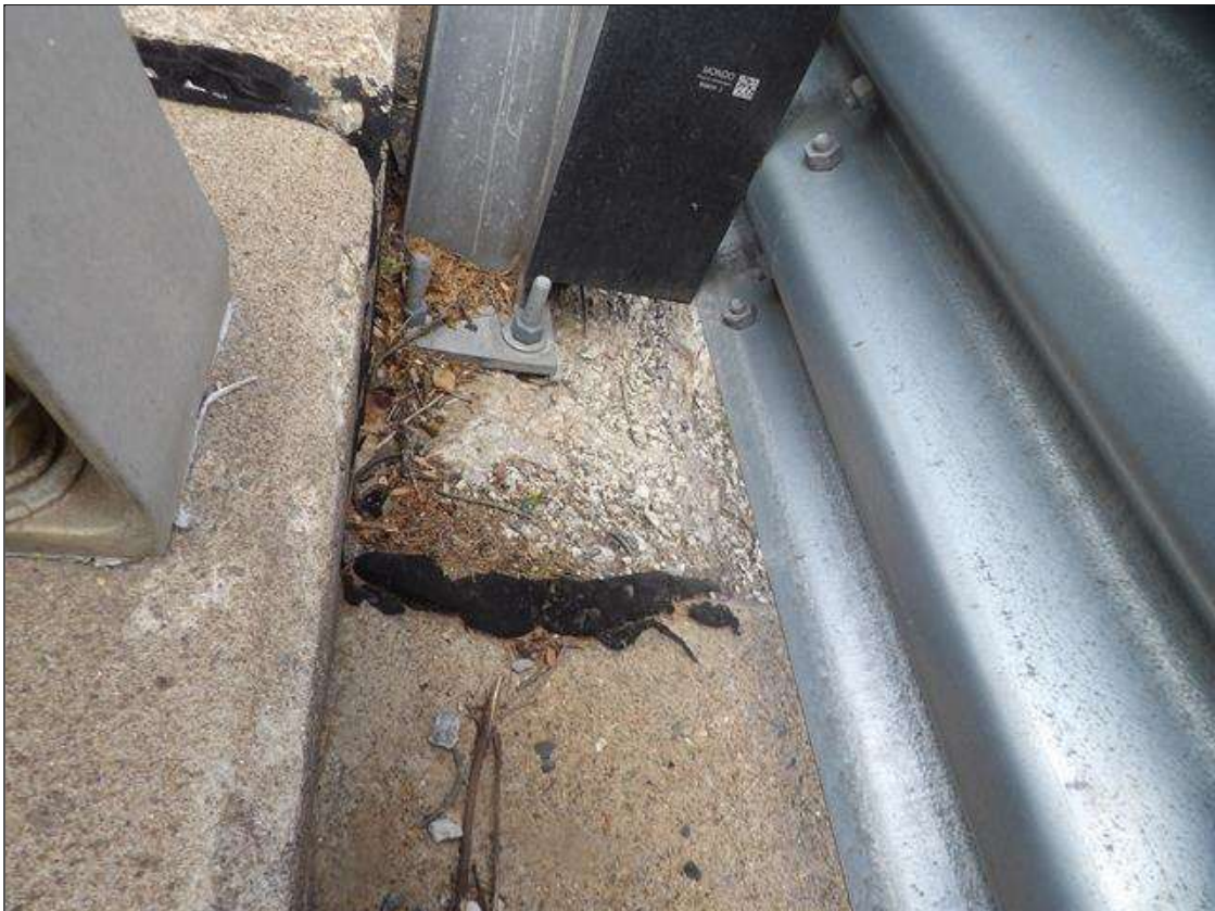
Span 4 Left Bridge Rail: SPALL WITH EXPOSED REBAR 8 INCHES WIDE X 18 INCHES LONG X 3 INCHES DEEP AT BENT 3
