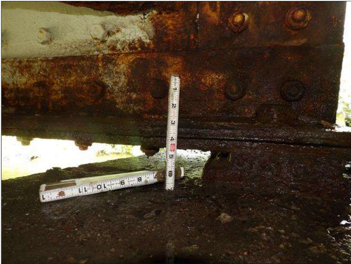
Span 2 Beam 1: AT BENT 2 END, REPAIR HAS BEEN INSTALLED CONSISTING OF 6 INCH X 6 INCH X 1/2 INCH ANGLE THAT IS 5 FEET LONG BOLTED TO WEB AND FLANGE WITH 3/4 INCH DIAMETER BOLTS SPACED AT 6 INCH ON CENTER. WEB HAS 10 INCH LONG X 1 FEET 9 INCH HIGH X 3/8 INCH THICK PLATE ALSO BOLTED WITH 3/4 INCH DIAMETER BOLTS. ANGLE HAS 1/16 INCH SECTION LOSS ON OUTER EDGES WITH 7/16 INCH AVERAGE REMAINING AND PLATE HAVE SURFACE CORROSION.
