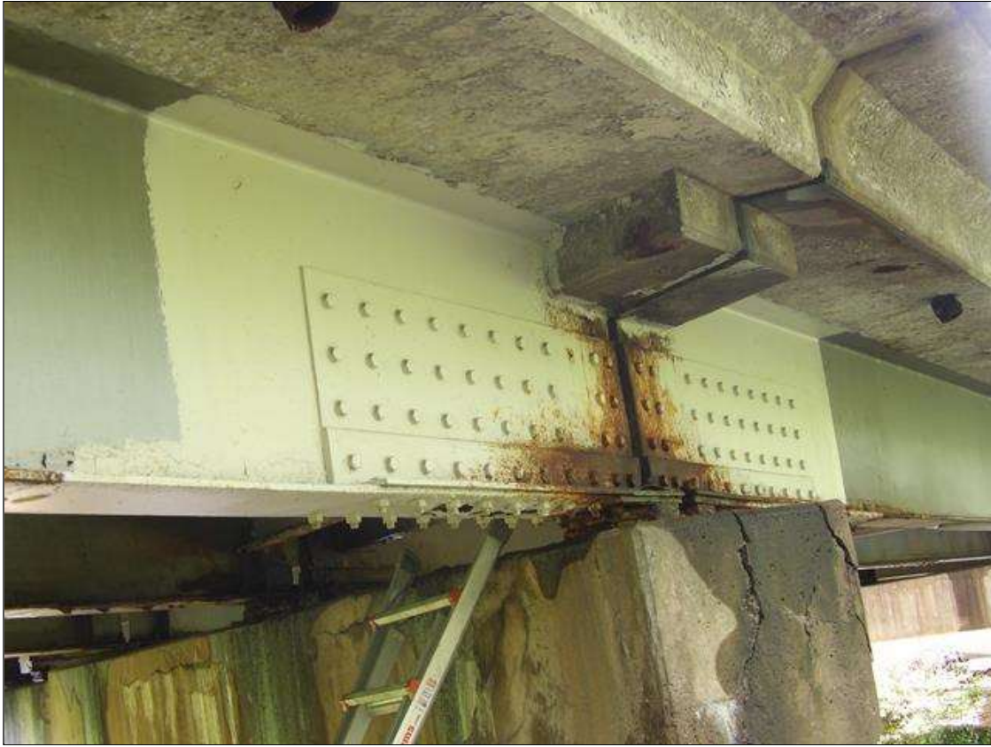
SPAN 3 BEAM 1 AT BENT 2 END, REPAIR PLATES 6 IN X 6 IN X 1/2 IN ANGLE THAT IS 5 FT LONG BOLTED TO WEB AND FLANGE WITH 3/4 IN DIAMETER BOLTS SPACED AT 6 IN ON CENTER. WEB HAS 10 IN LONG X 1 FT 9 IN HIGH X 3/8 IN THICK PLATE ALSO BOLTED WITH 3/4 IN DIAMETER BOLTS. ANGLE AND PLATE HAVE SURFACE RUST.
