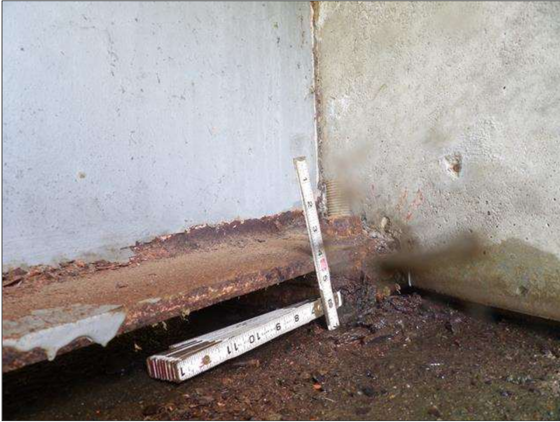
Span 4 Beam 4: CORROSION WITH 1/16 INCH LOSS OF SECTION ALONG RIGHT EDGE OF BOTTOM FLANGE WITH 9/16 INCH REMAINING 6 INCHES LONG X 2 INCHES WIDE AT END BENT 2
