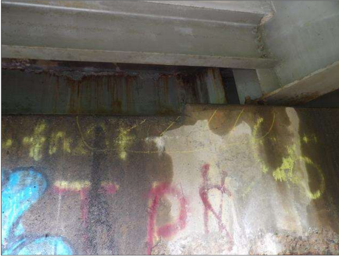
Bent 3 Cap 1: 36 INCHES X 6 INCHES X 12 INCHES AREA OF DELAMINATION WITH UP TO 1/32 INCHES LONGITUDINAL AND HORIZONTAL CRACKS IN TOP AND SPAN 4 FACE OF CAP BENEATH BAY 3
