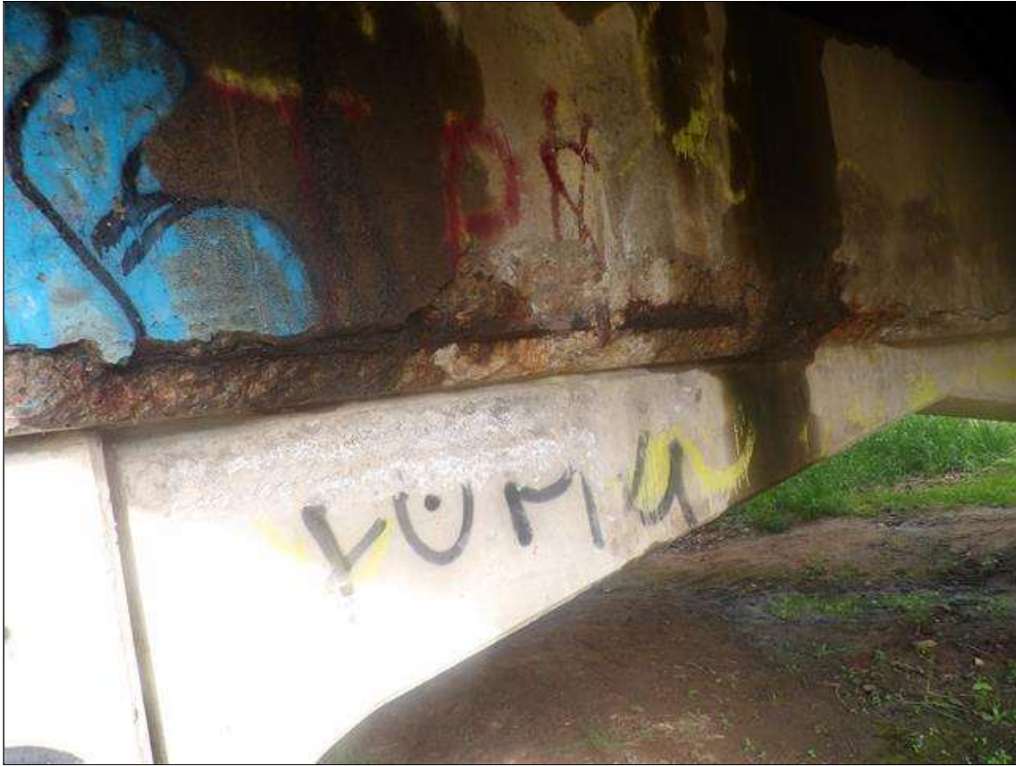
Bent 3 Cap 1: PAR: 96 INCHES X 6 INCHES X 9 INCHES SPALL WITH EXPOSED REBAR WITH MINOR SECTION LOSS AND 125 INCHES X 6 INCHES X 12 INCHES AREA OF DELAMINATION WITH UP TO 1/4 INCHES LONGITUDINAL AND HORIZONTAL CRACKS IN BOTTOM AND SPAN 4 FACE OF CAP BETWEEN COLUMNS
