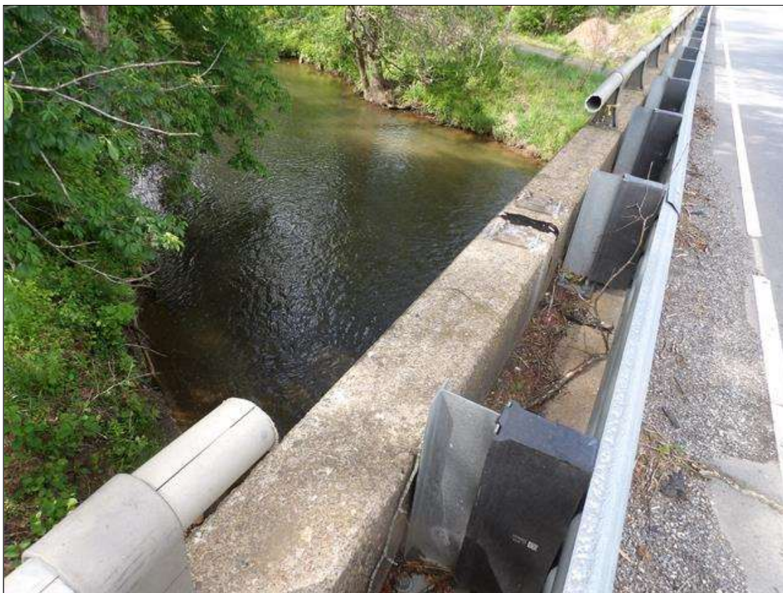
Span 2 Left Bridge Rail: 15 FEET SECTION OF IMPACT DAMAGE WITH SEPARATED, CRACKED AND MISSING RAIL AND RAIL POSTS EXTENDING FROM BENT 1; CONDITION MITIGATED WITH ADDITION OF THREE BEAM METAL RAIL
