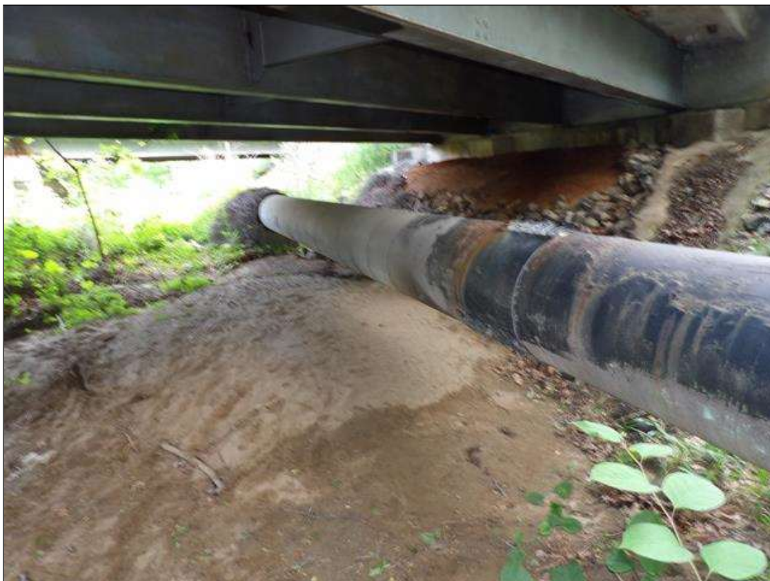
UTILITY UNDER SPAN 1, NOT ATTACHED TO BRIDGE
