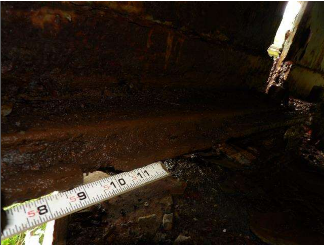
Span 3 Beam 4: PAR--6 FOOT LONG CORROSION IN BOTTOM FLANGE REPAIR PLATE WITH 1/4 INCH AVERAGE REMAINING WITH 1 1/2 INCH X 1/2 INCH HOLE IN LEFT SIDE AT 18 INCHES FROM BEARING, BOTTOM FLANGE BELOW REPAIR PLATE WITH 3/8 INCH AVERAGE REMAINING WITH 24 INCH X UP TO 1 1/2 INCH WIDE HOLE IN LEFT SIDE STARTING AT BEARING. MEASUREMENTS OF WELDED PLATE REPAIRS ON BOTH FACES OF WEB AND BOTTOM FLANGE UP TO 60 INCHES LONG X 21 1/2 INCHES HIGH X 1/2 INCH THICK IN WEB, AND 60 INCHES LONG X 4 INCHES WIDE X 1/2 INCH THICK IN FLANGE AT BENT 2
