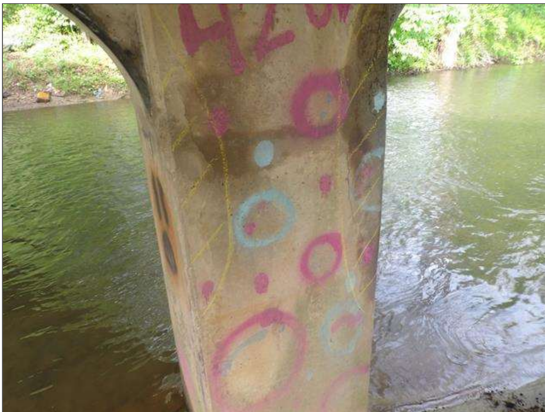
Bent 2 Pile 1: (2) AREAS OF DELAMINATION UP TO 36 INCHES X 7 INCHES X 5 INCHES WITH 1/16 INCHES VERTICAL CRACKS IN NORTHWEST AND NORTHEAST CORNERS OF COLUMN, APPROXIMATELY 3 FEET FROM BOTTOM OF CAP
