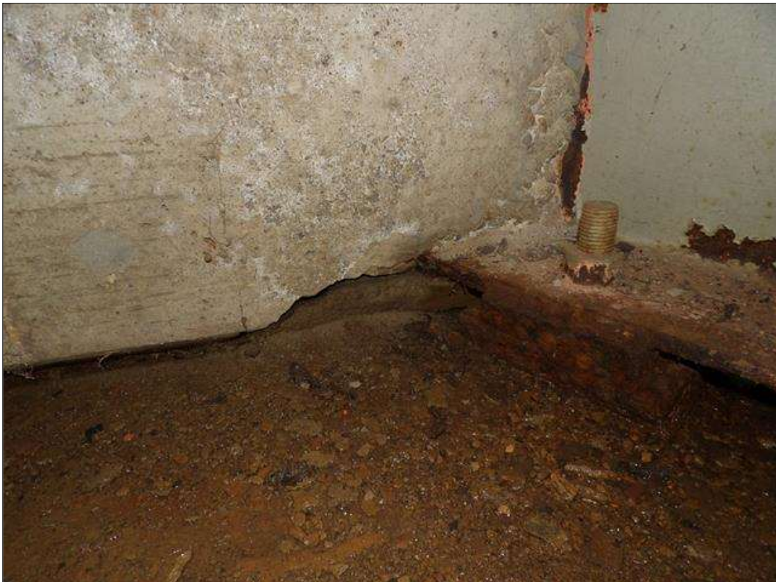
End Bent 1 Abutment: UP TO 6 INCH X 2 INCH X 1/4 INCH DEEP SPALL IN FACE OF CURTAIN WALL RIGHT EDGE OF BOTTOM FLANGE OF BEAMS 1 AND 3
