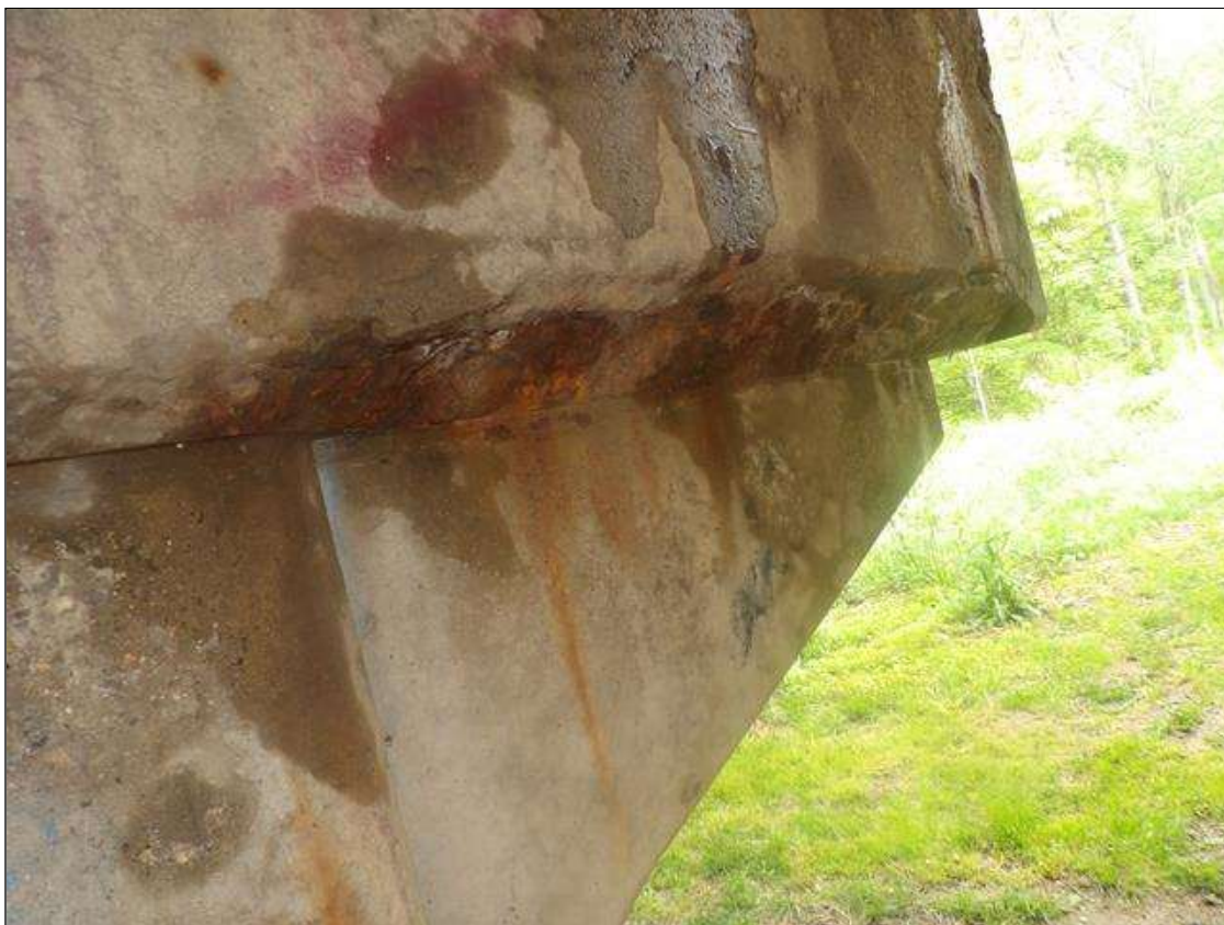
Bent 3 Cap 1: 60 INCHES X 6 INCHES X 4 INCHES SPALL WITH EXPOSED REBAR NO LOSS IN BOTTOM AND SPAN 4 FACE OF CAP AT LEFT END
