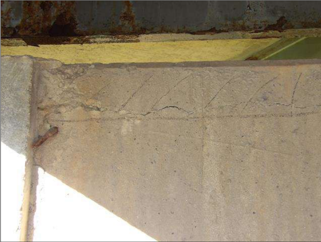
Bent 3 Cap 1: 32 INCHES X 9 INCHES X 7 INCHES AREA OF DELAMINATION WITH UP TO 1/16 INCHES HORIZONTAL CRACKS IN TOP AND SPAN 4 FACE OF CAP TO LEFT OF BEAM 4
