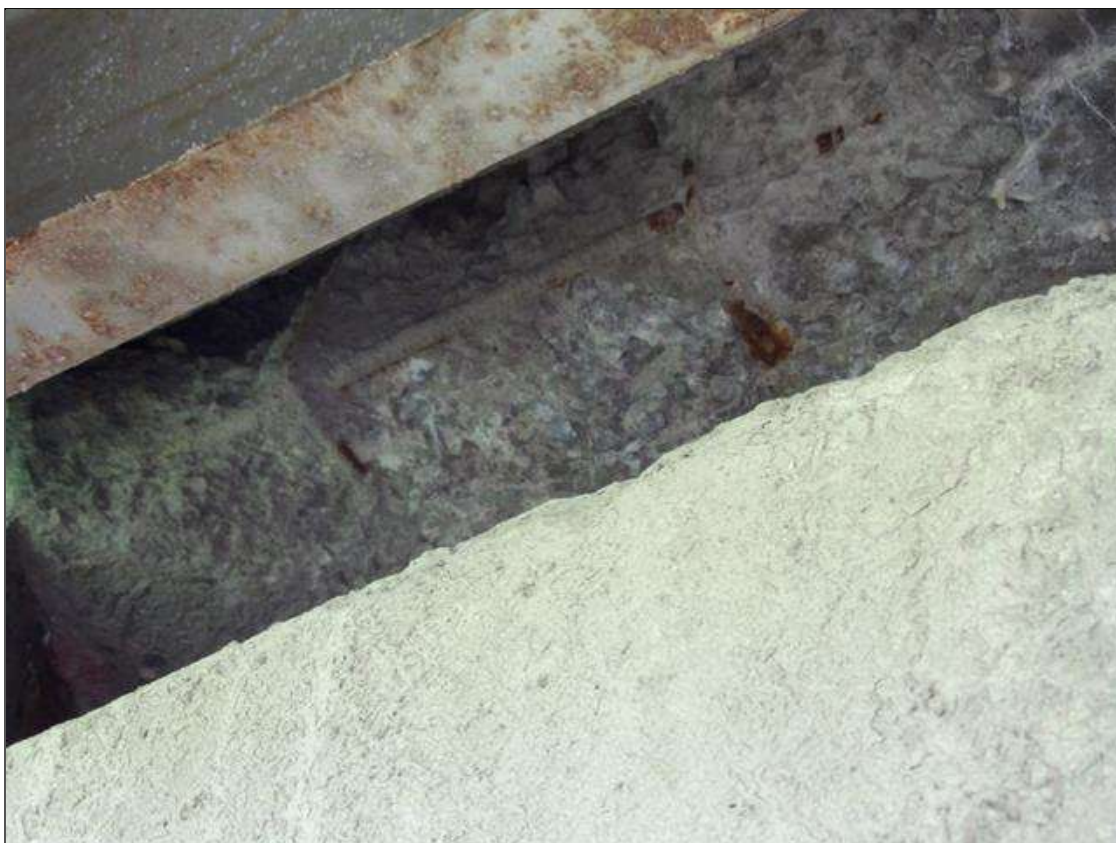
TYPICAL DIAPHRAGM SPALL WITH EXPOSED REBAR NO LOSS, BAY 3 SPAN 3 AT PIER 2 SHOWN
