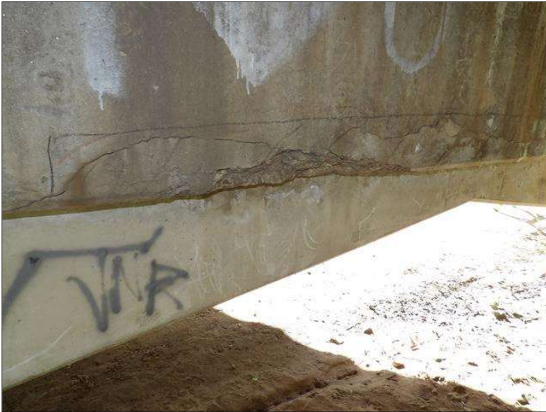
Bent 3 Cap 1: 90 INCHES X 6 INCHES X 8 INCHES AREA OF DELAMINATION WITH UP TO 1/16 INCHES LONGITUDINAL AND HORIZONTAL CRACKS AND 32 INCHES X 4 INCHES X 4 INCHES SPALL IN BOTTOM AND SPAN 3 FACE OF CAP, BEGINNING APPROXIMATELY 3 FEET TO RIGHT OF COLUMN 1
