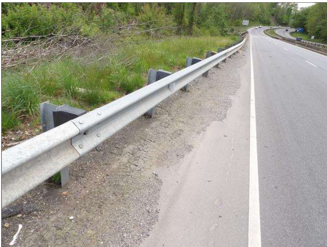
NORTHEAST GUARDRAIL HAS BEEN REPLACED 50 FOOT LONG 50 FOOT FROM BRIDGE
