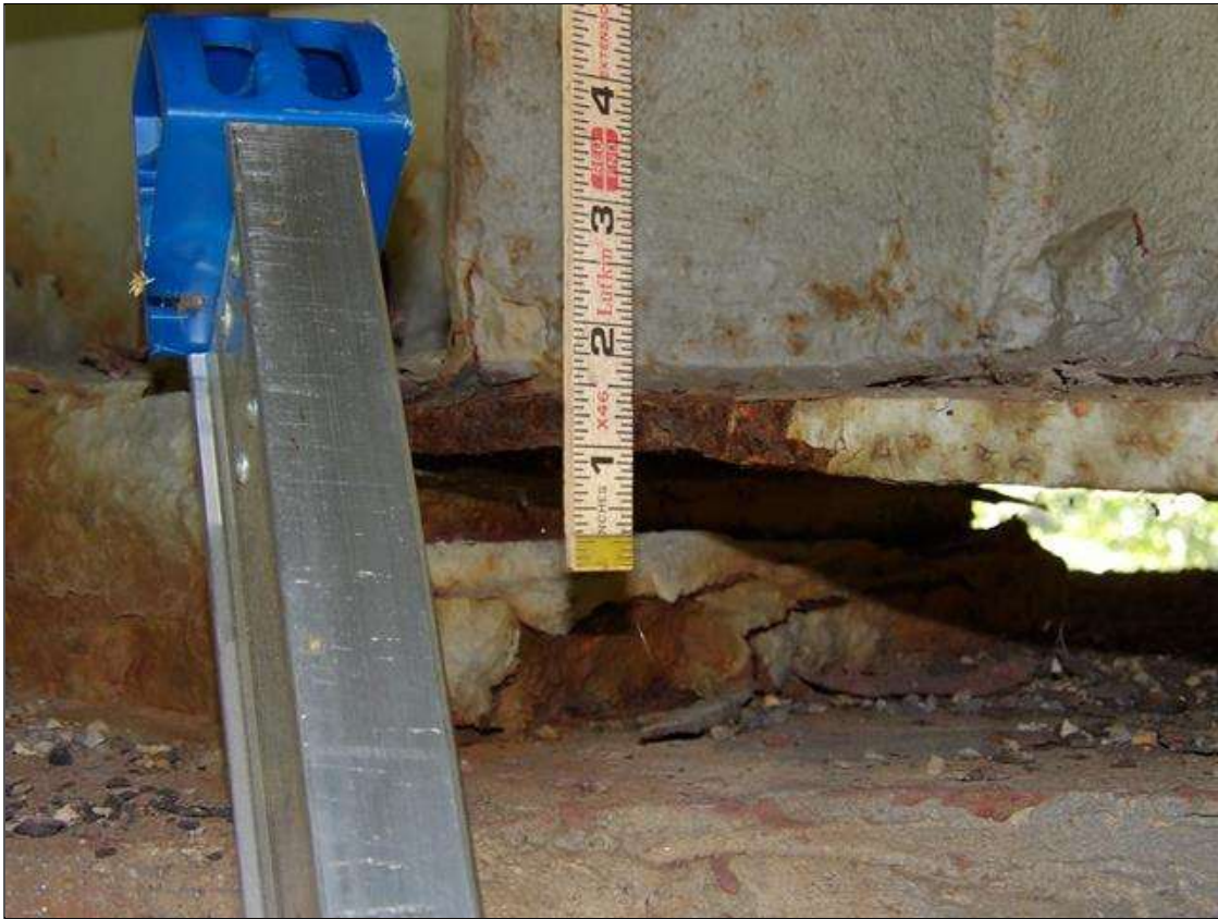
Span 1 Beam 2: PAR: CORROSION ALONG BOTTOM FLANGE 8 INCHES LONG X 11 1/2 INCHES WIDE DOWN TO 3/8 INCHES RESIDUAL THICKNESS AT BENT 1
