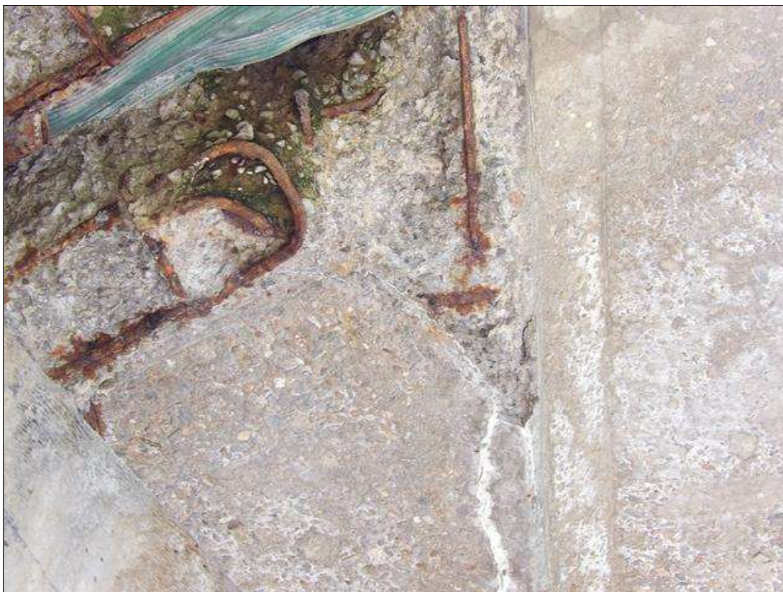
Span 2 Deck: PAR: 26 INCHES X 14 INCHES X 4 INCHES DEEP SPALL WITH EXPOSED REBAR WITH MINOR LOSS IN BOTTOM OF RIGHT OVERHANG ABOVE BENT 1
