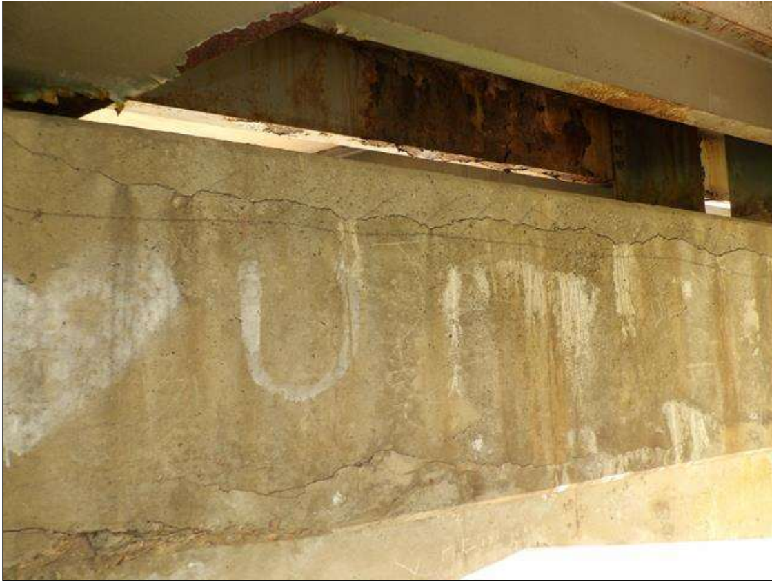
Bent 3 Cap 1: 10 FEET X 8 INCHES X 10 INCHES AREA OF DELAMINATION WITH UP TO 1/8 INCHES HORIZONTAL CRACKS WITH AND WITHOUT EFFLORESCENCE IN TOP AND SPAN 3 FACE OF CAP BENEATH BAY 2
