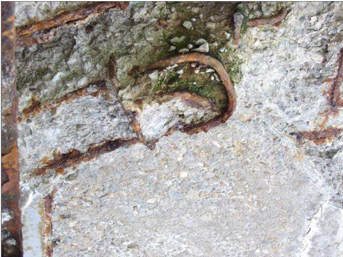
PAR-- SPAN 2 BENT 1 RIGHT OVERHANG DIAPHRAGM, SPALL 1 FEET LONG X 2 FEET WIDE X FULL DEPTH WITH EXPOSED REBAR WITH 60 PERCENT SECTION LOSS
