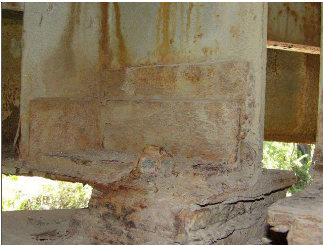
SPAN 2 BEAM 3--WELDED REPAIR PLATE LEFT SIDE AT PIER 1 BOTTOM FLANGE ANGLE 12 INCH LONG X 4 INCH X 4 INCH X 1/2 INCH, WEB 12 INCH LONG X 6 INCH HIGH X 1/4 INCH , STIFFNER 4 INCH X 4 INCH X 1/2 AT BOTTOM
