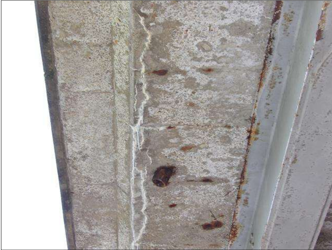
Span 2 Deck: UP TO 1/32 INCHES TRANSVERSE AND LONGITUDINAL CRACKS WITH EFFLORESCENCE AND RUST STAINING THROUGHOUT BOTTOM OF RIGHT OVERHANG IN VARIOUS LOCATIONS
