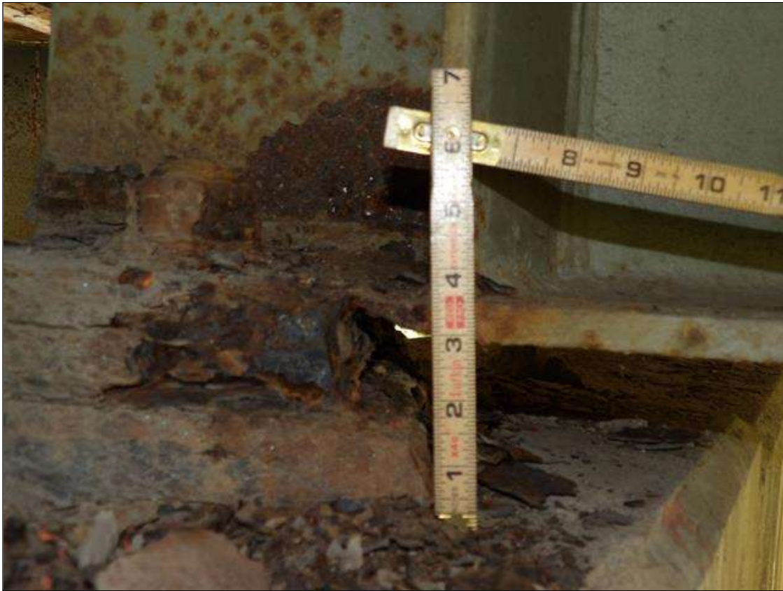
Span 1 Beam 3: PAR: CORROSION ALONG BOTH FACES OF WEB AND BOTTOM FLANGE UP TO 10 INCHES LONG X 6 INCHES HIGH DOWN TO 1/2 INCHES RESIDUAL WEB, WEB HAS A 1 INCH X 1/16 INCH PERFORATION OVER BEARING AND 9 INCHES LONG X 11 1/2 INCHES WIDE DOWN TO 1/4 INCHES RESIDUAL FLANGE WITH 1/4 INCH VERTICAL DEFORMATION IN BOTTOM FLANGE AT BEARING PLATE AT BENT 1
