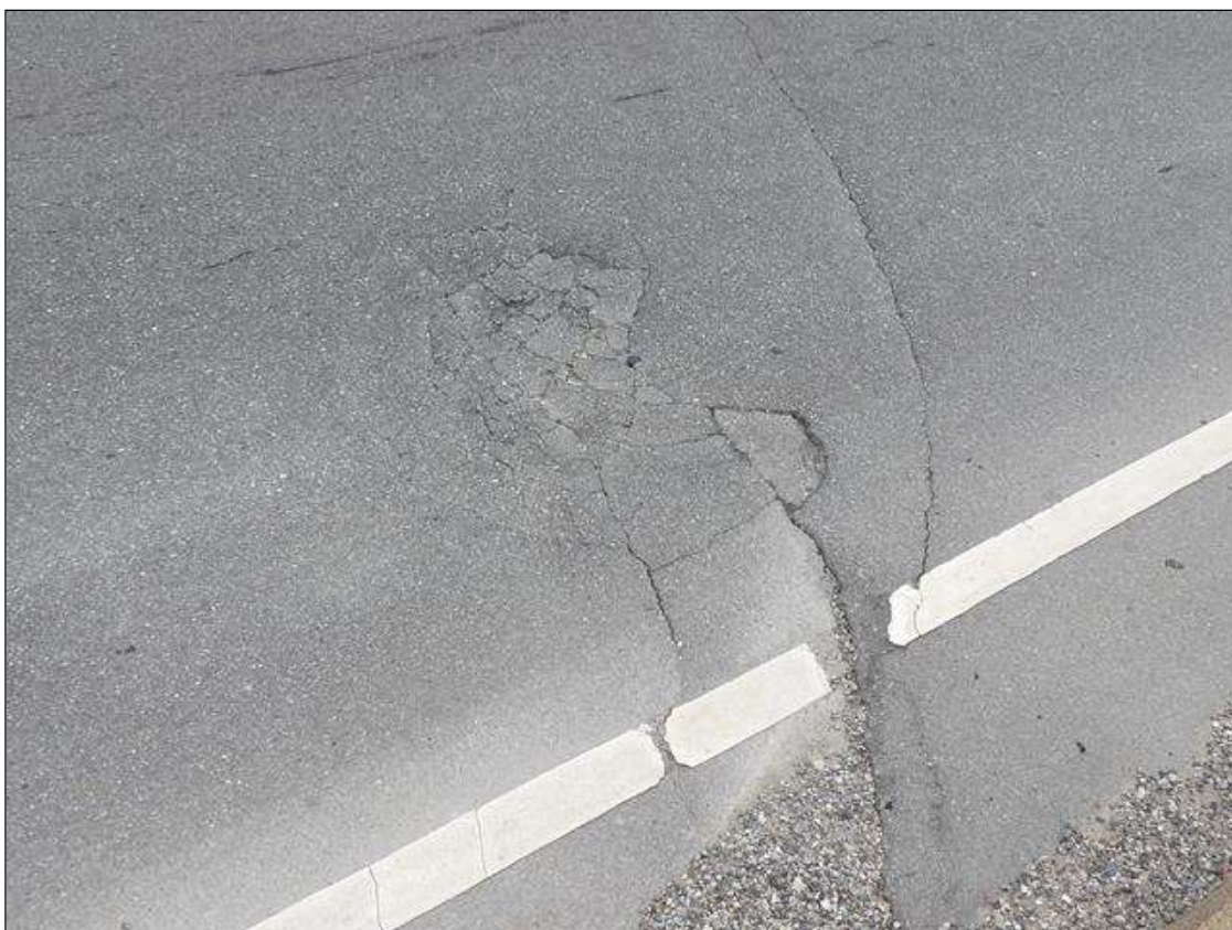
Span 2 Wearing Surface: 4 FOOT X 2 FOOT AREA OF DETERIORATED ASPHALT IN RIGHT LANE AT PIER 2
