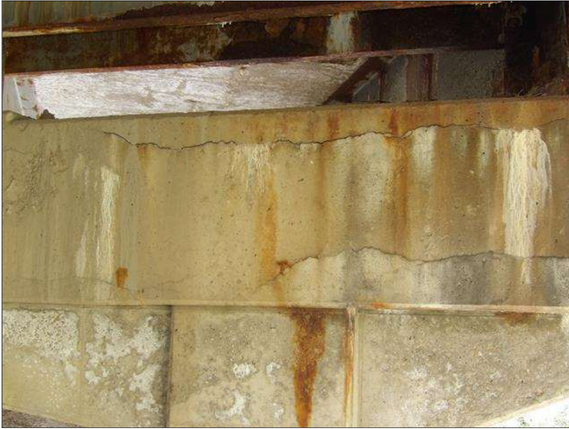
Bent 1 Cap 1: UP TO 3/8 INCHES LONGITUDINAL AND HORIZONTAL CRACKS WITH AND WITHOUT EFFLORESCENCE AND AREAS OF DELAMINATION THROUGHOUT TOP, BOTTOM AND SPAN 1 FACE OF CAP FROM BEAM 3 TO RIGHT END
