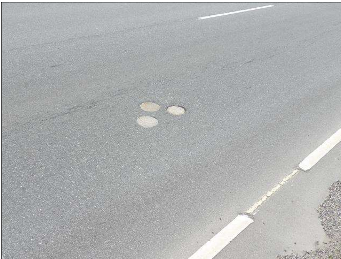
Span 3 Wearing Surface: (3) 8 INCHES DIAMETER FILLED CORED HOLES IN OUTSIDE LANE NEAR MIDSPAN
