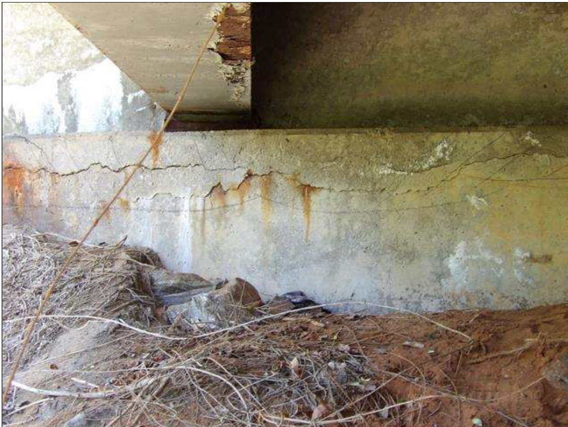
End Bent 1 Cap 1: 10 FEET X 9 INCHES X 13 INCHES AREA OF DELAMINATION WITH UP TO 1/4 INCHES LONGITUDINAL AND HORIZONTAL CRACKS IN TOP AND FACE OF CAP BENEATH BEAM 4 AND BAY 3
