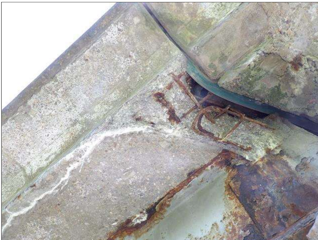
Span 2 Deck: 30 INCHES X 18 INCHES X 4 INCHES DEEP SPALL WITH EXPOSED REBAR NO LOSS IN BOTTOM OF RIGHT OVERHANG ABOVE BENT 2
