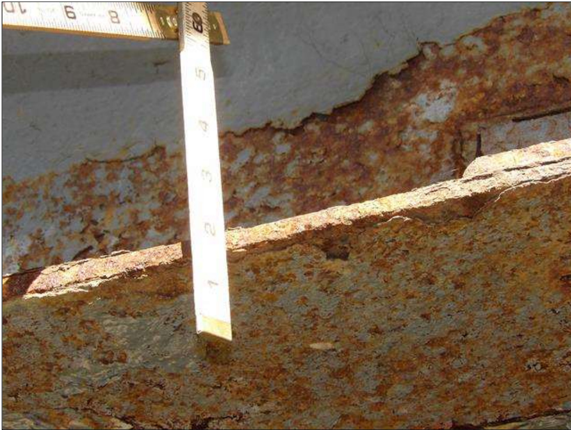
Span 3 Beam 4: PAR: CORROSION ALONG RIGHT FACE OF WEB AND BOTTOM FLANGE UP TO 60 INCHES LONG X 6 INCHES HIGH DOWN TO 1/2 INCHES RESIDUAL WEB, AND 48 INCHES LONG X 5 1/2 INCHES WIDE DOWN TO 3/8 INCHES RESIDUAL FLANGE, EXTENDING FROM PLATE REPAIR 1 FEET FROM BENT 3
