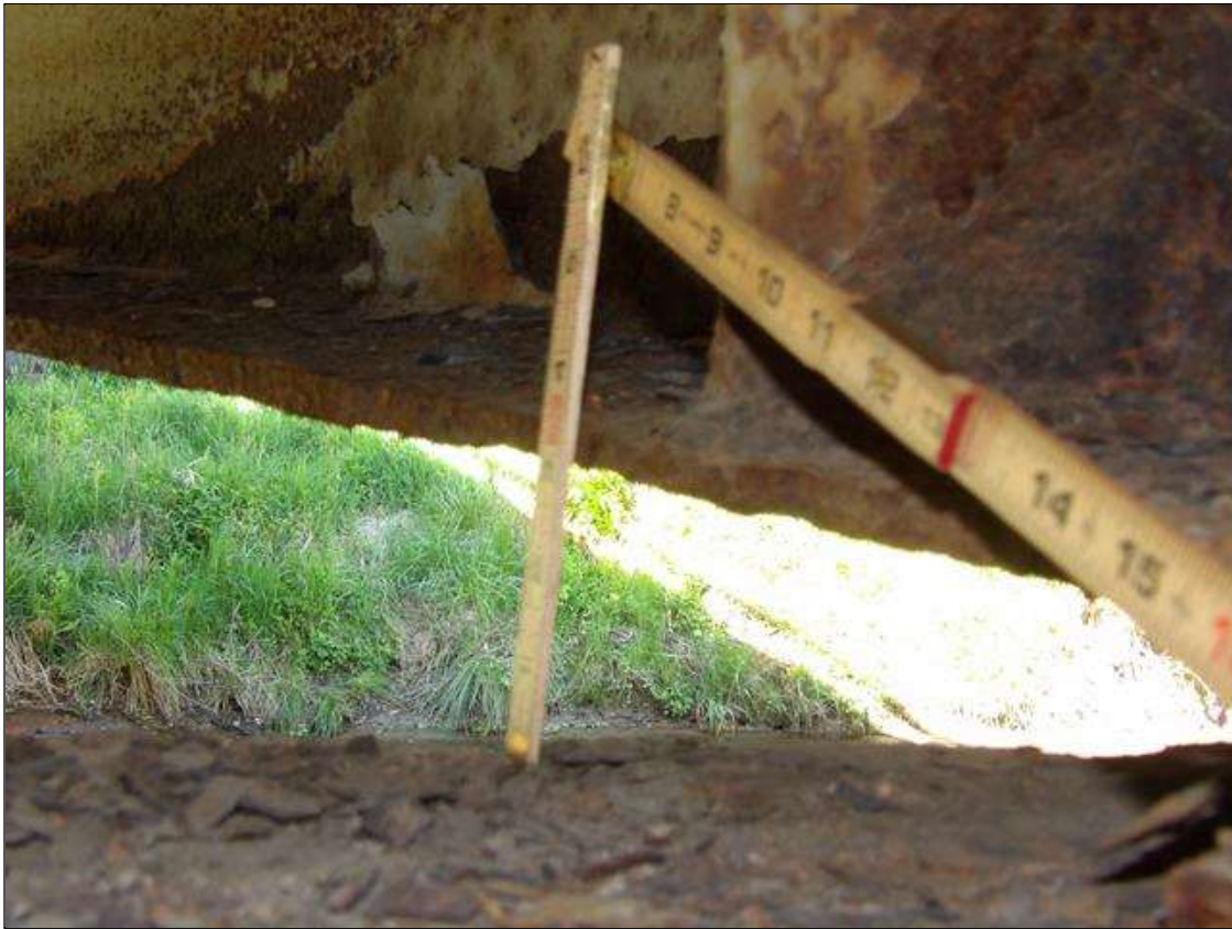
Span 2 Beam 2: PAR: CORROSION ALONG BOTH FACES OF WEB AND BOTTOM FLANGE UP TO 48 INCHES LONG X 10 INCHES HIGH DOWN TO 1/2 INCHES RESIDUAL WEB, AND 48 INCHES LONG X 11 1/2 INCHES WIDE DOWN TO 3/8 INCHES RESIDUAL FLANGE AT BENT 2
