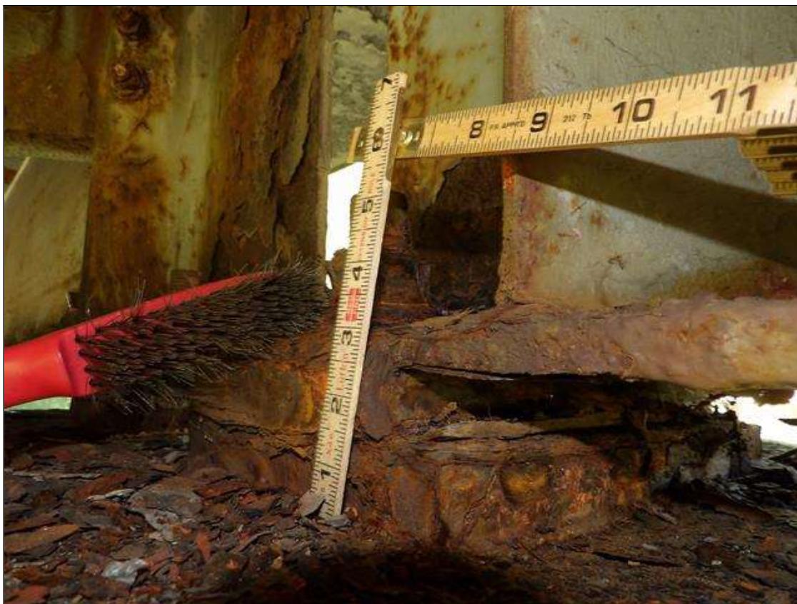
Span 3 Beam 1: CORROSION ALONG BOTH FACES OF WEB AND BOTTOM FLANGE UP TO 5 FEET LONG X 6 INCHES HIGH DOWN TO 1/2 INCHES RESIDUAL WEB, AND 5 FEET LONG X 11 1/2 INCHES WIDE DOWN TO 1/2 INCHES RESIDUAL FLANGE AT BENT 2
