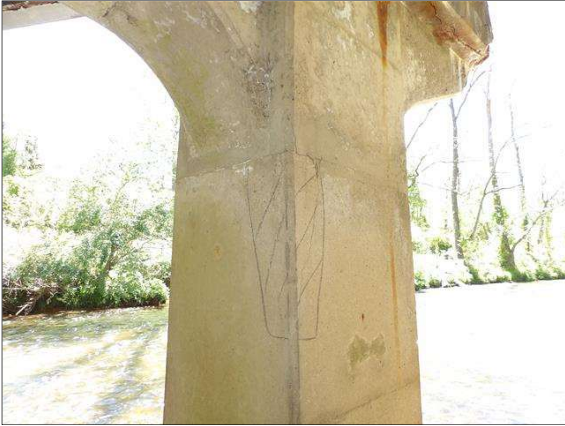
Bent 1 Pile 2: 33 INCHES X 6 INCHES X 9 INCHES AREA OF DELAMINATION WITH UP TO 1/16 INCHES VERTICAL CRACKS IN SOUTHWEST CORNER OF COLUMN, APPROXIMATELY 3 FEET FROM BOTTOM OF CAP
