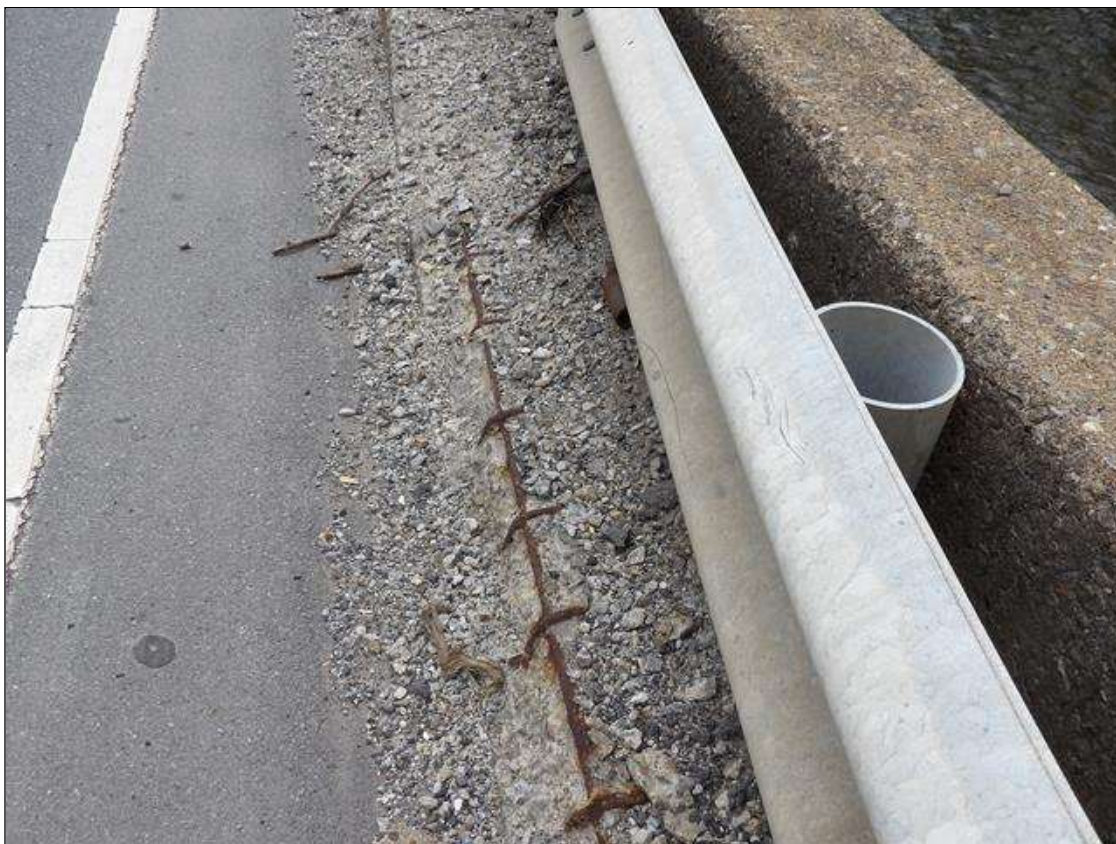
Span 1 Right Bridge Rail: RIGHT CURB HAS DETERIORATED CONCRETE ON TOP AND VERTICAL FACES 18 IN WIDE UP TO 2.5 IN DEEP WITH REBAR EXPOSED WITH ONSET OF SECTION LOSS AT BEGINNING 30 FEET OF SPAN
