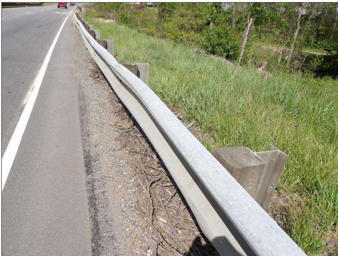
SOUTHEAST GUARDRAIL IMPACT DAMAGE 10 FOOT LONG 50 FEET FROM BRIDGE
