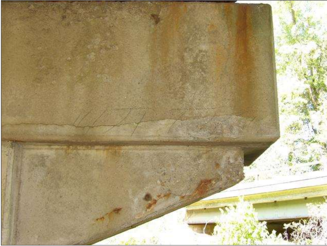
Bent 2 Cap 1: 55 INCHES X 4 INCHES X 10 INCHES AREA OF DELAMINATION WITH UP TO 1/16 INCHES LONGITUDINAL AND HORIZONTAL CRACKS IN BOTTOM AND SPAN 3 FACE OF CAP AT LEFT END
