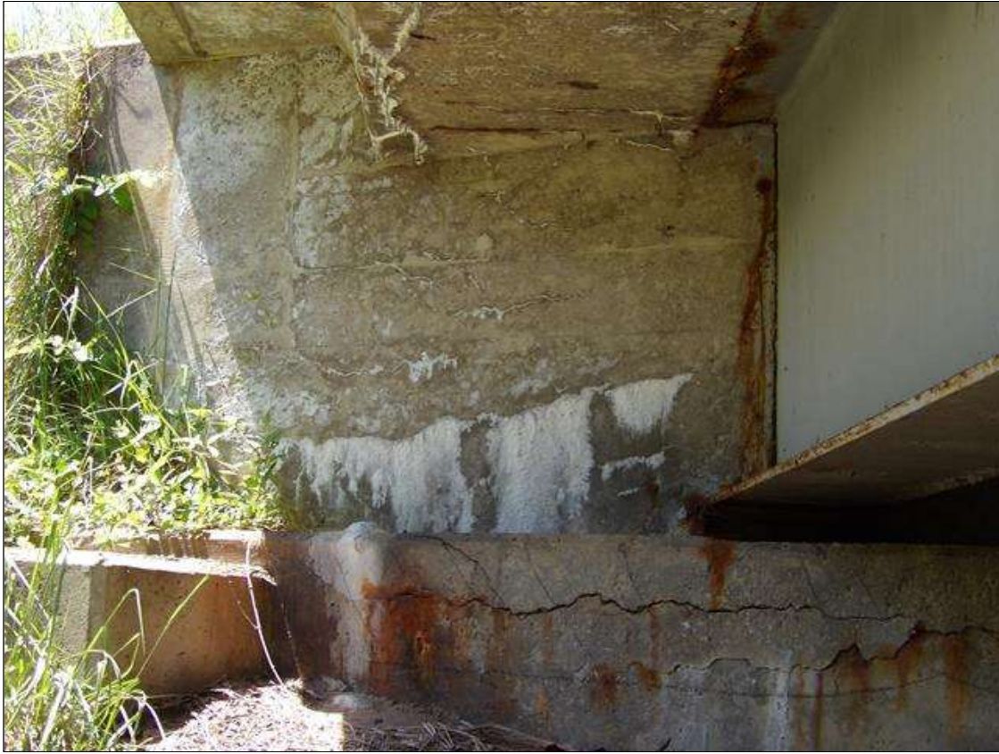
End Bent 1 Abutment: 57 INCHES X 42 INCHES AREA OF HAIRLINE HORIZONTAL AND MAP CRACKS WITH EFFLORESCENCE IN FACE OF CURTAIN WALL AT RIGHT END
