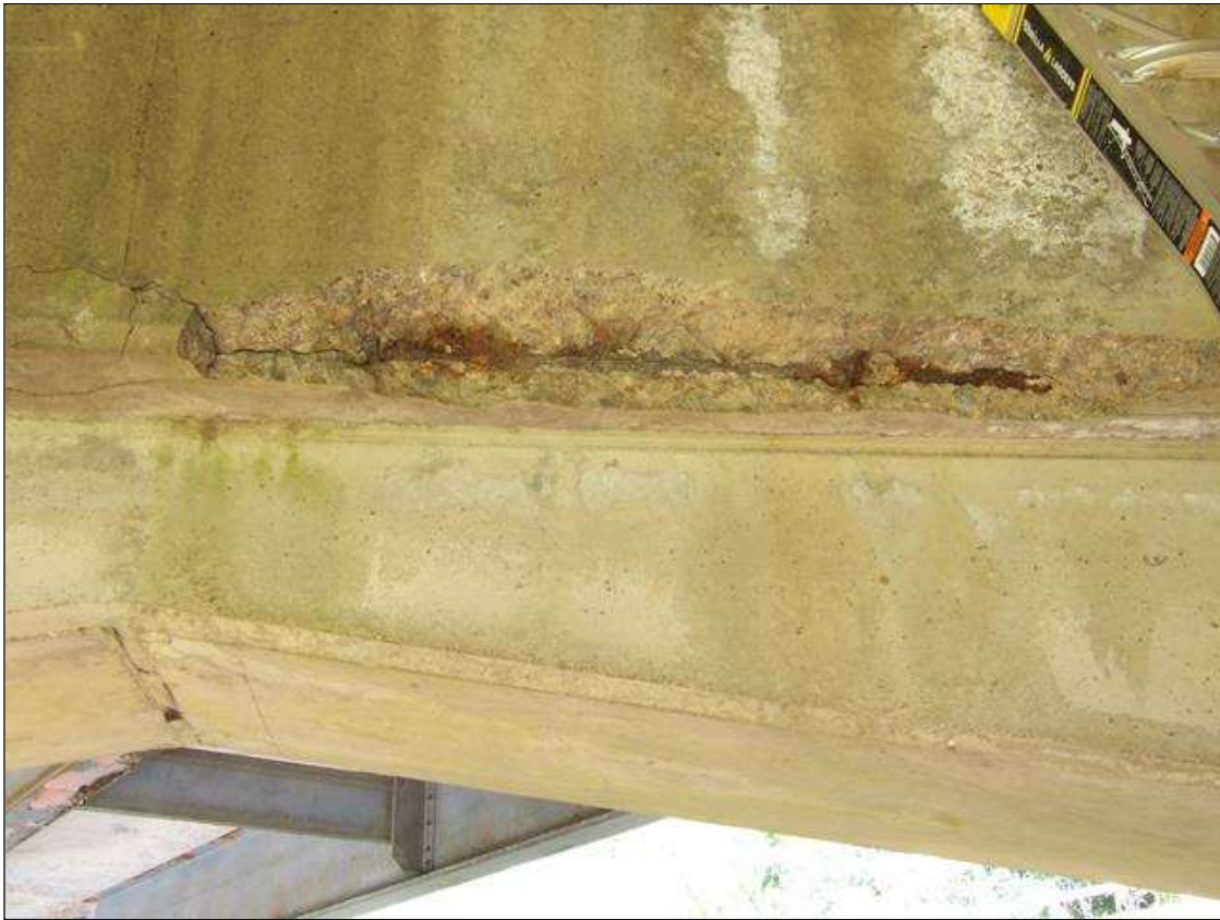
Bent 2 Cap 1: 51 INCHES X 6 INCHES X 10 INCHES AREA OF DELAMINATION WITH UP TO 0.035 INCHES LONGITUDINAL AND HORIZONTAL CRACKS AND 40 INCHES X 6 INCHES X 2 INCHES DEEP SPALL WITH EXPOSED REBAR NO LOSS IN BOTTOM AND SPAN 3 FACE OF CAP TO RIGHT OF COLUMN 1
