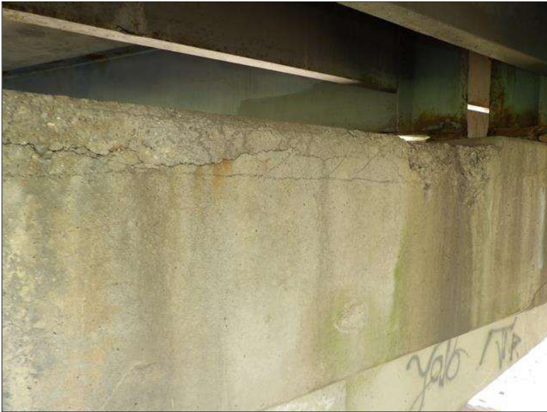
Bent 3 Cap 1: 9 FEET X 30 INCHES X 30 INCHES AREA OF DELAMINATION WITH 3/8 INCHES LONGITUDINAL AND HORIZONTAL CRACKS WITH AND WITHOUT EFFLORESCENCE, AND (2) SPALLS UP TO 28 INCHES X 12 INCHES X 10 INCHES IN TOP AND BOTH FACES OF CAP FROM LEFT END TO BAY 2 SOUTH FACE SHOWN
