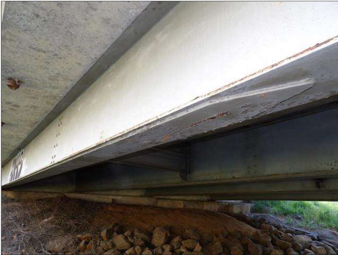
Span 1 Beam 4: SPOT FRECKLED SURFACE RUST ON WEB AND FLANGES.
