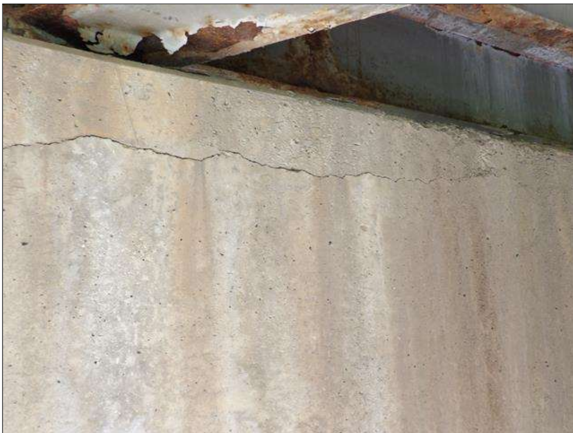
Bent 3 Cap 1: UP TO 1/16 INCHES HORIZONTAL CRACKS WITH AREAS OF DELAMINATION UP TO 50 INCHES X 7 INCHES X 6 INCHES IN TOP, BOTTOM AND SPAN 4 FACE OF CAP BENEATH BAY 2 AND BEAM 3
