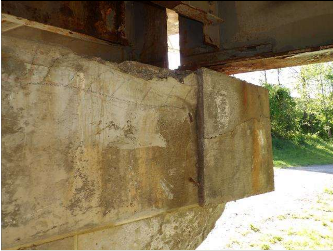
Bent 3 Cap 1: 70 INCHES X 8 INCHES X 9 INCHES AREA OF DELAMINATION WITH UP TO 1/16 INCHES LONGITUDINAL AND HORIZONTAL CRACKS WITH AND WITHOUT EFFLORESCENCE, AND 32 INCHES X 9 INCHES X 9 INCHES UNSOUND PATCH WITH 15 INCHES X 5 INCHES X 1 INCHES DEEP SPALL IN TOP AND SPAN 3 FACE OF CAP BENEATH BAY 3 AND BEAM 4
