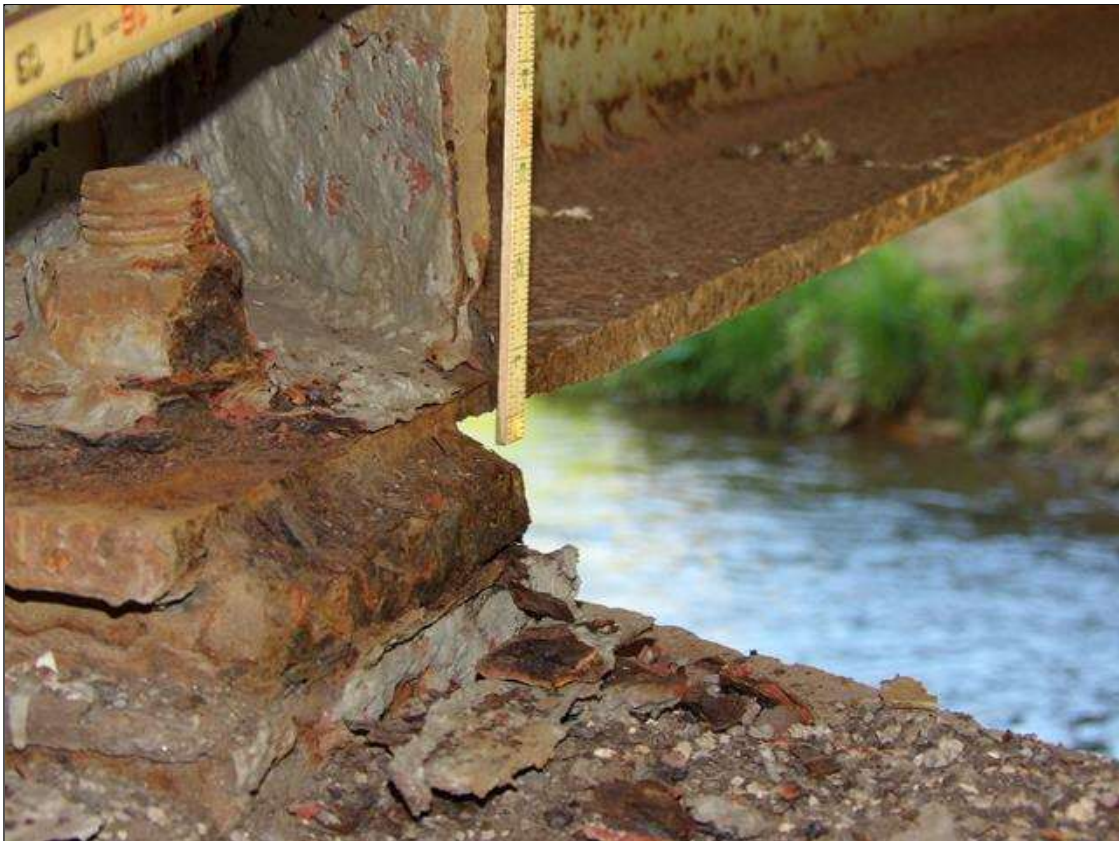
Span 2 Beam 2: PAR: CORROSION ALONG BOTTOM FLANGE 10 INCHES LONG X 11 1/2 INCHES WIDE DOWN TO 5/16 INCHES RESIDUAL THICKNESS ON RIGHT SIDE AT BENT 1
