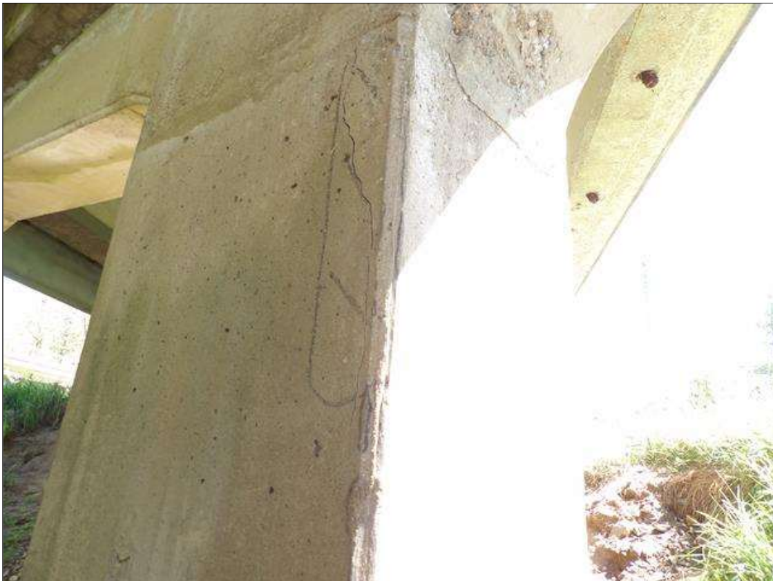
Bent 2 Pile 2: 32 INCHES HIGH UP TO 1/16 INCHES VERTICAL CRACK IN SOUTHEAST CORNER OF COLUMN, APPROXIMATELY 3 FEET FROM BOTTOM OF CAP
