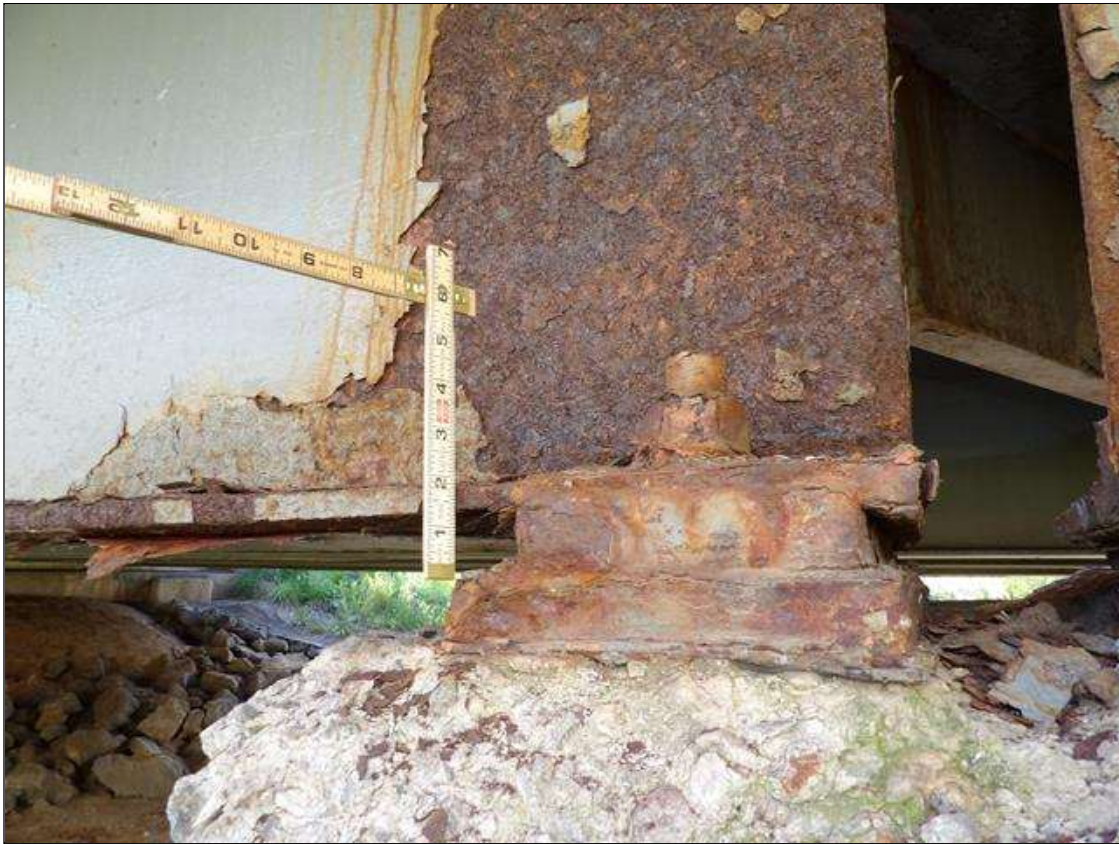
Span 4 Beam 1: CORROSION ALONG BOTH FACES OF WEB AND BOTTOM FLANGE UP TO 29 INCHES LONG X 31 1/2 INCHES HIGH DOWN TO 1/2 INCHES RESIDUAL WEB, AND 36 INCHES LONG X 11 1/2 INCHES WIDE DOWN TO 1/2 INCHES RESIDUAL FLANGE AT BENT 3
