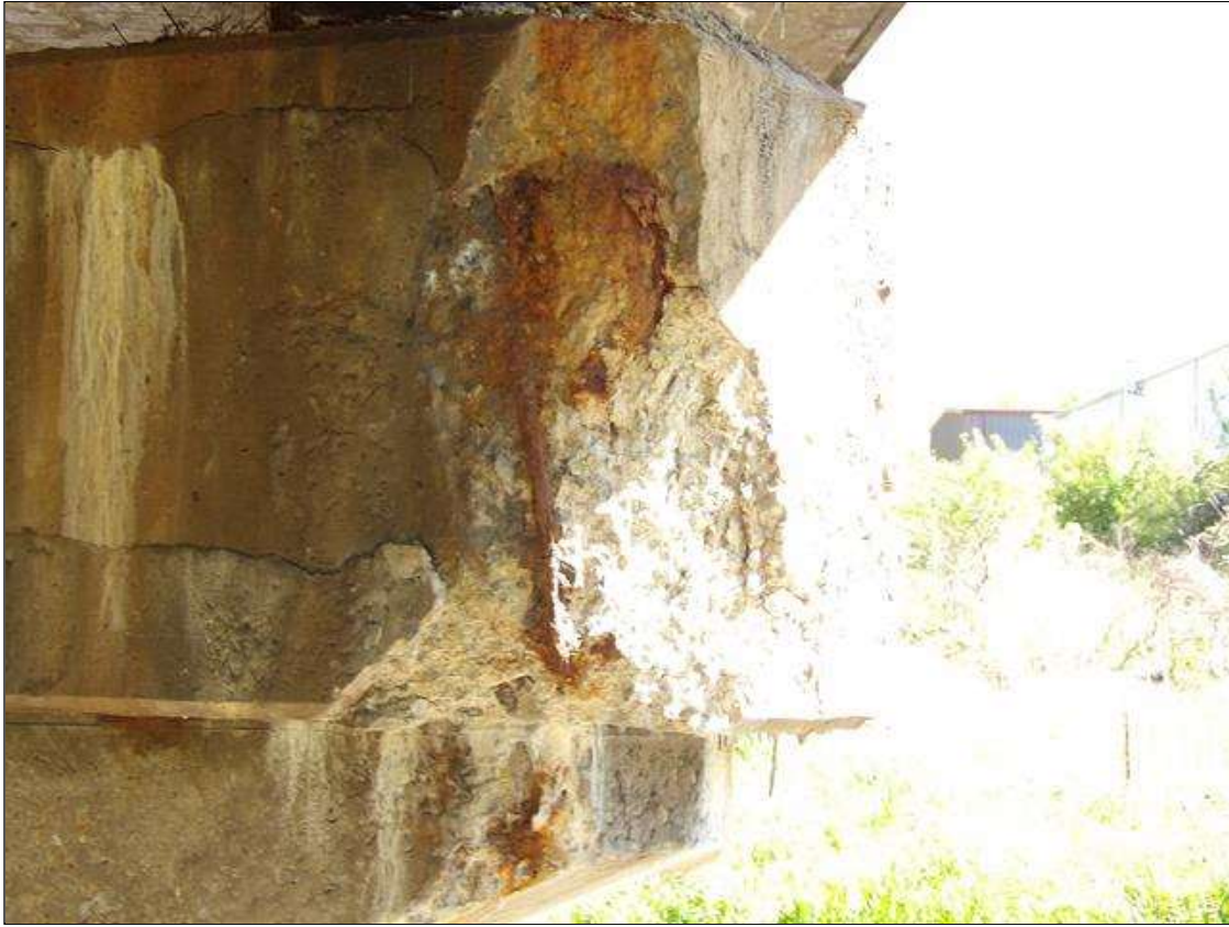
Bent 1 Cap 1: PAR: 30 INCHES X 12 INCHES X 6 INCHES DEEP SPALL WITH EXPOSED REBAR WITH SECTION LOSS IN SPAN 1 FACE OF CAP AT RIGHT END
