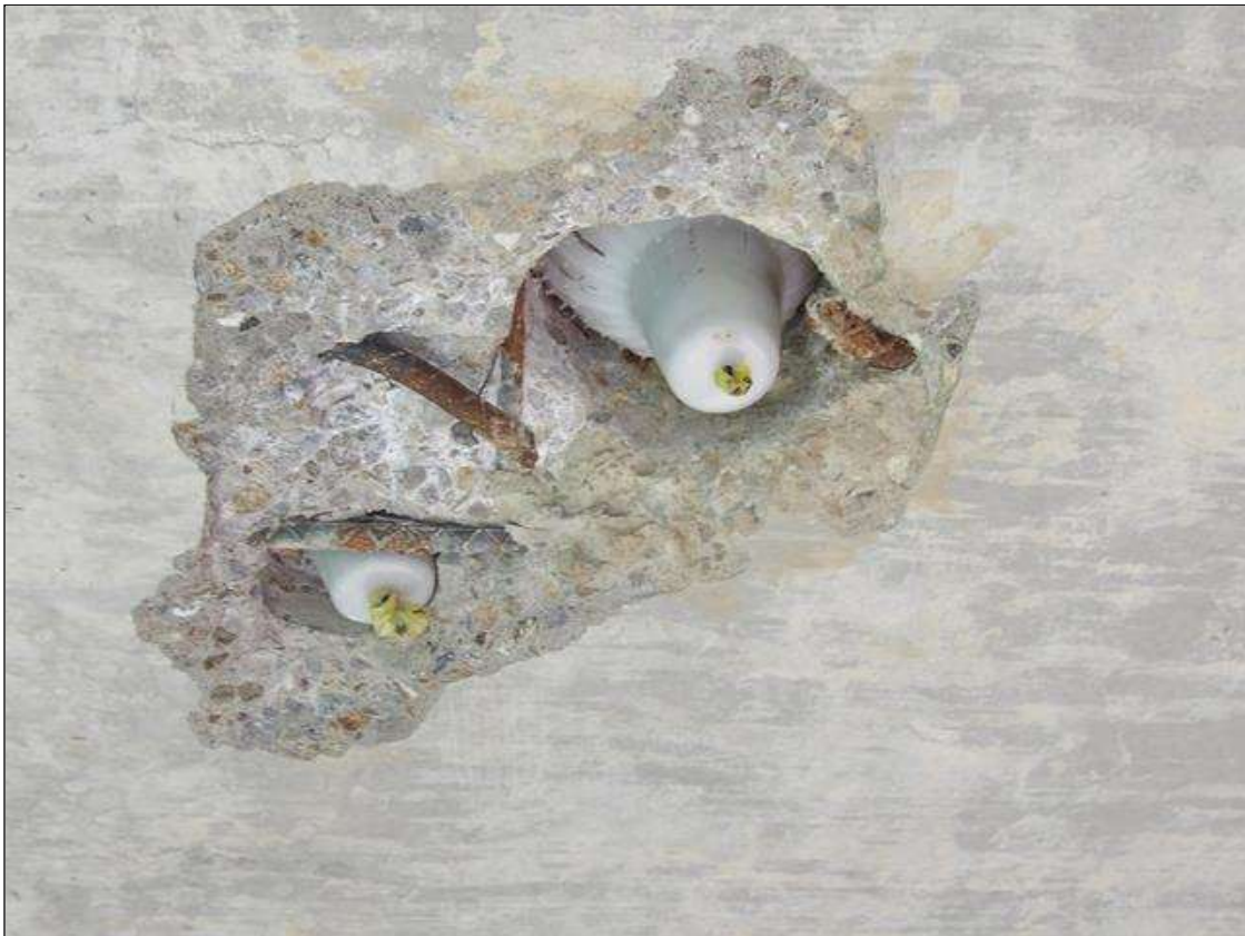
Span 3 Deck: PAR--23 INCHES X 19 INCHES X 6 INCHES DEEP SPALL WITH EXPOSED BROKE REBAR DUE TO CORE IN BOTTOM OF DECK AT CORE HOLE LOCATIONS IN BAY 3 NEAR MIDSPAN
