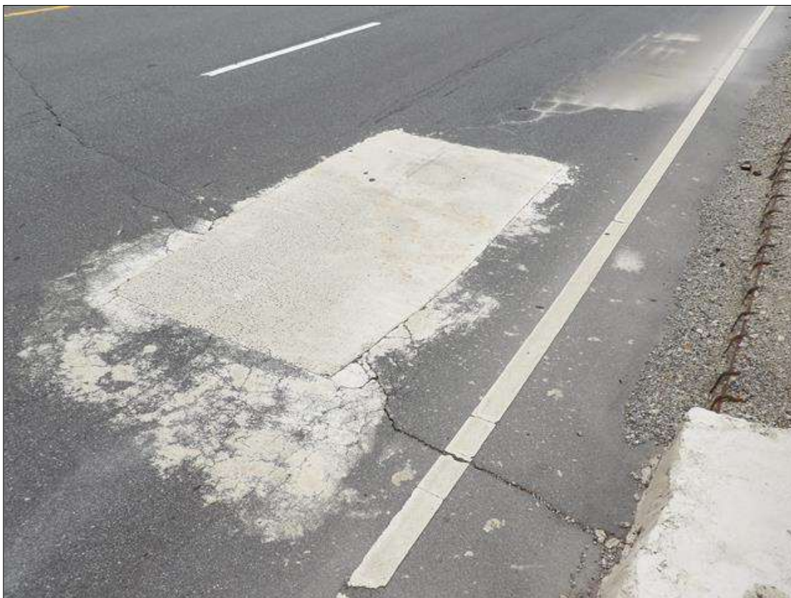
Span 2 Wearing Surface: SOUND PATCH 5 FOOT X 3 FOOT IN RIGHT TRAVEL LANE OVER PIER 1
