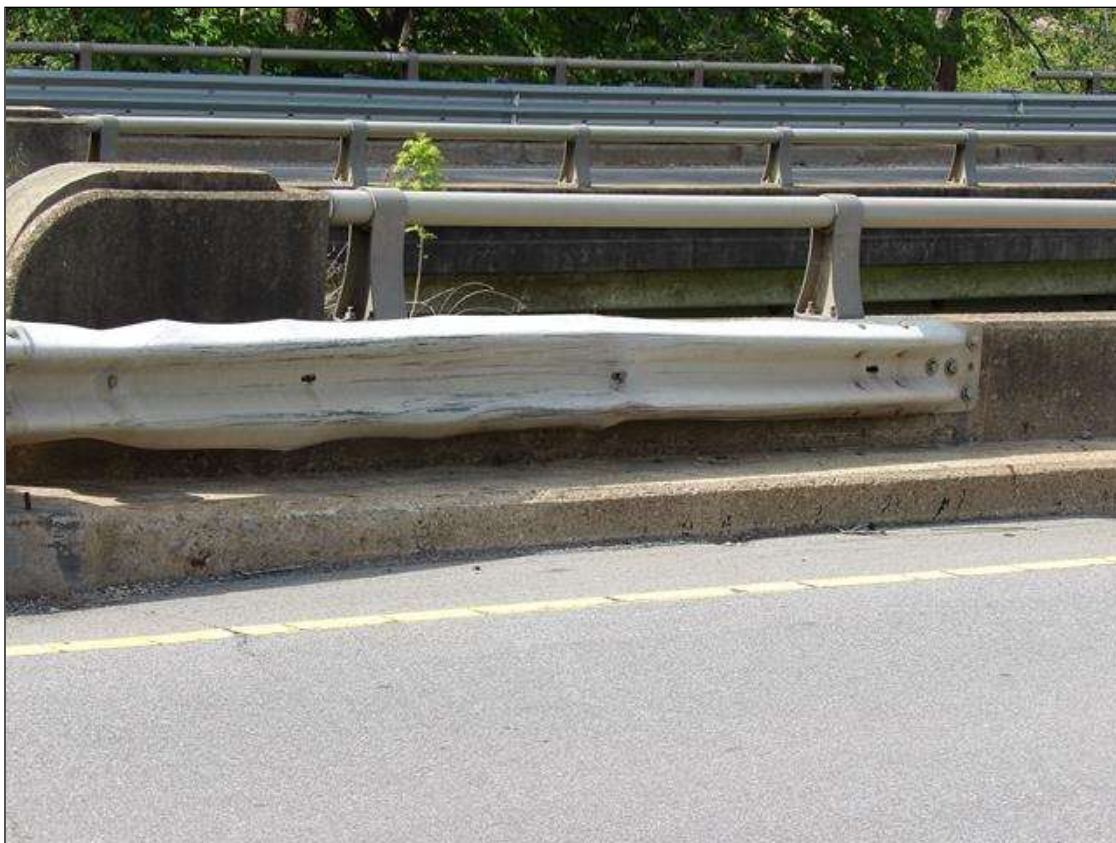
SOUTHWEST GUARDRAIL IMPACT DAMAGE 10 FOOT LONG AT BRIDGE
