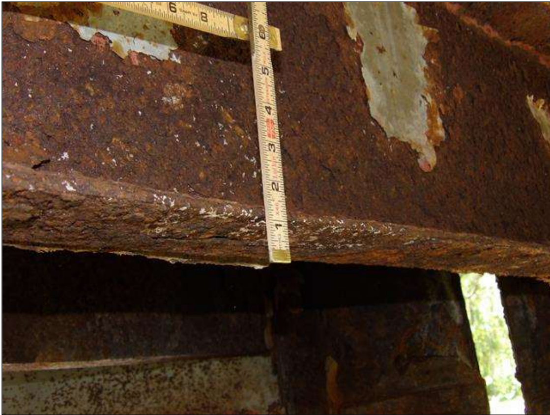
Span 1 Beam 4: PAR: CORROSION THROUGHOUT BENT 1 DIAPHRAGM UP TO 6 FEET LONG X 14 INCHES HIGH DOWN TO 1/4 INCHES RESIDUAL WEB, AND 6 FEET LONG X 3 1/2 INCHES WIDE DOWN TO 1/4 INCHES RESIDUAL FLANGES IN BAY 3
