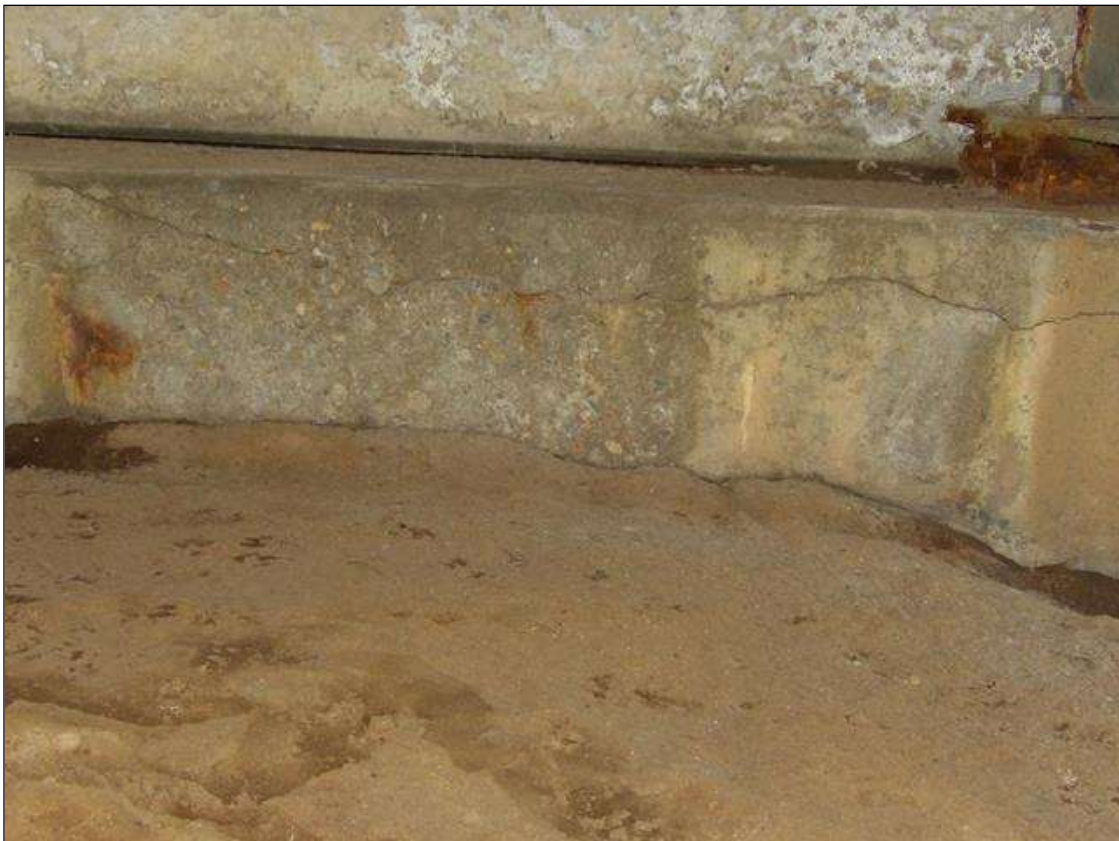
End Bent 2 Cap 1: BELOW BAY 3, 11 FEET LONG X UP TO 1/8 INCH WIDE HORIZONTAL CRACK
