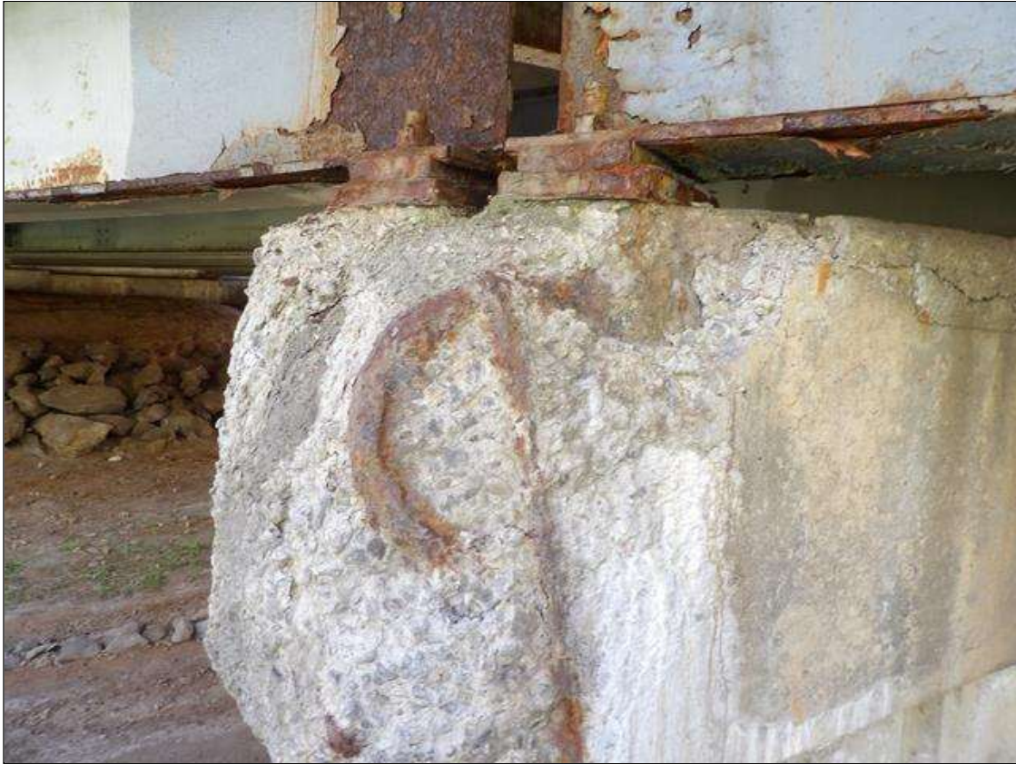
Bent 3 Cap 1: PAR: 26 INCHES X 20 INCHES X 30 INCHES SPALL WITH EXPOSED REBAR IN LEFT END OF CAP WITH MINOR LOSS OF BEARING LESS THAN 5 PERCENT UNDER BOTH BEARINGS
