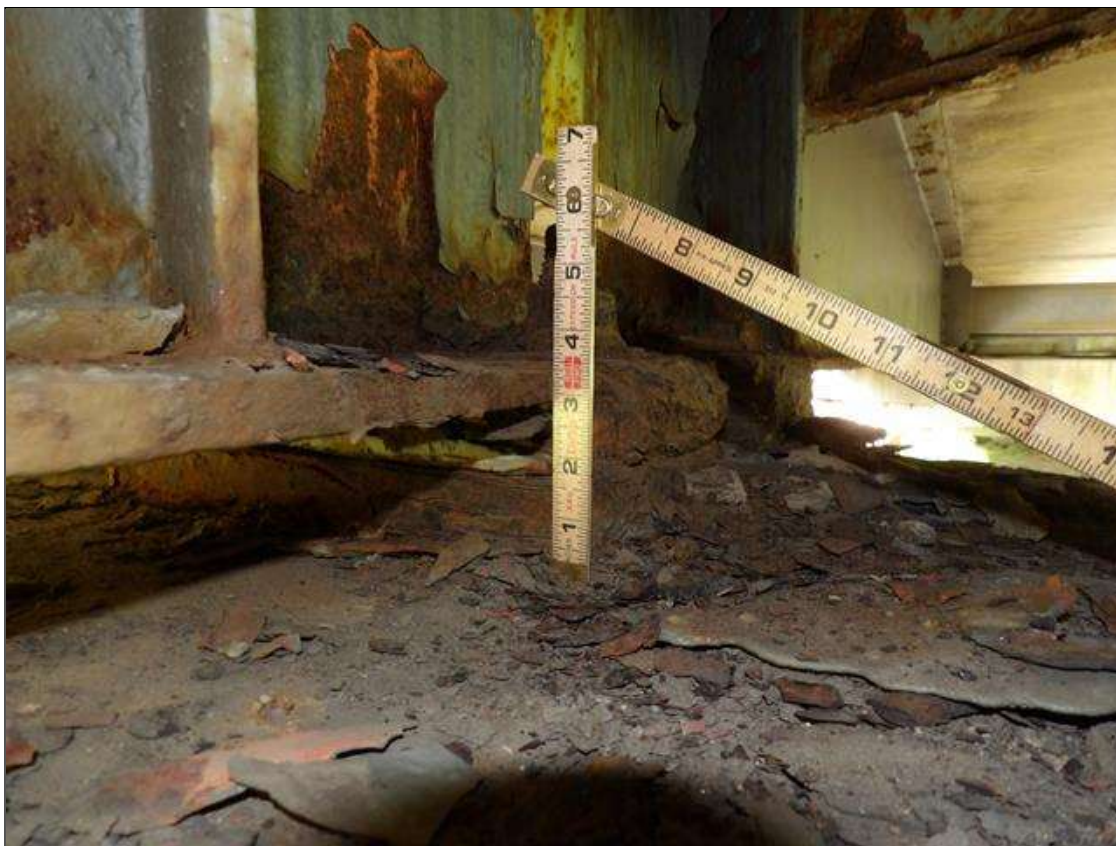
Span 3 Beam 3: PAR: CORROSION ALONG BOTH FACES OF WEB AND BOTTOM FLANGE UP TO 11 INCHES LONG X 4 INCHES HIGH DOWN TO 1/2 INCHES RESIDUAL WEB, AND 12 INCHES LONG X 5 1/2 INCHES WIDE DOWN TO 3/8 INCHES RESIDUAL FLANGE AT BENT 2
