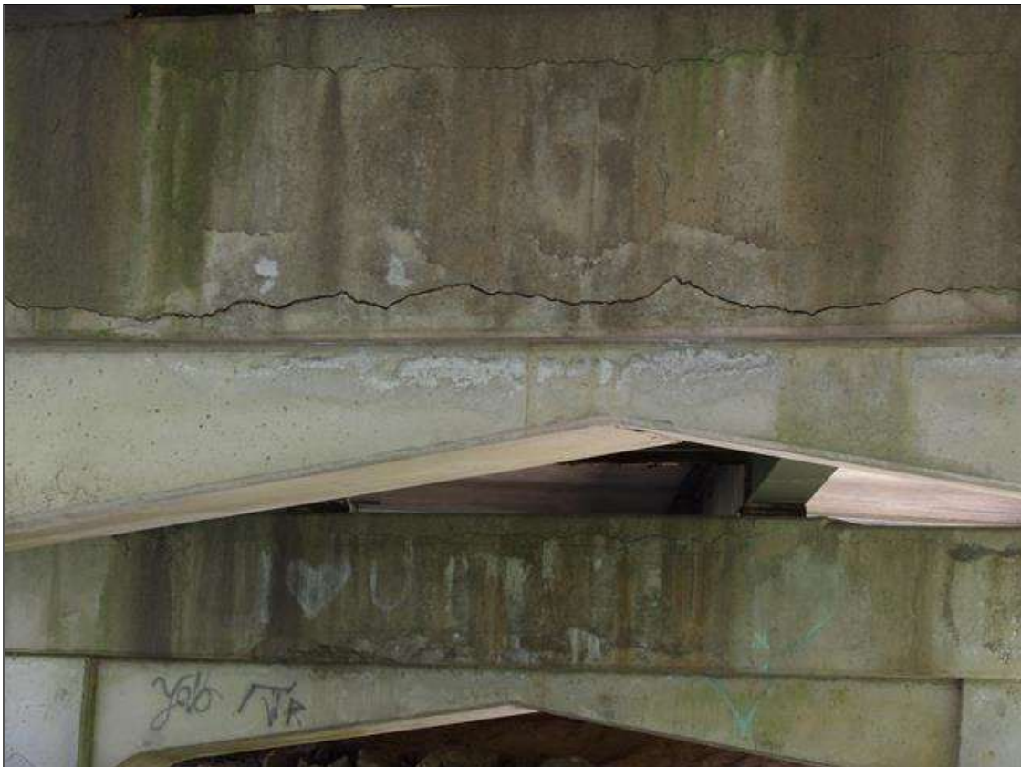
Bent 2 Cap 1: 31 FEET OF UP TO 3/8 INCHES LONGITUDINAL AND HORIZONTAL CRACKS WITH AND WITHOUT EFFLORESCENCE AND AREAS OF DELAMINATION THROUGHOUT TOP, BOTTOM AND SPAN 2 FACE OF CAP
