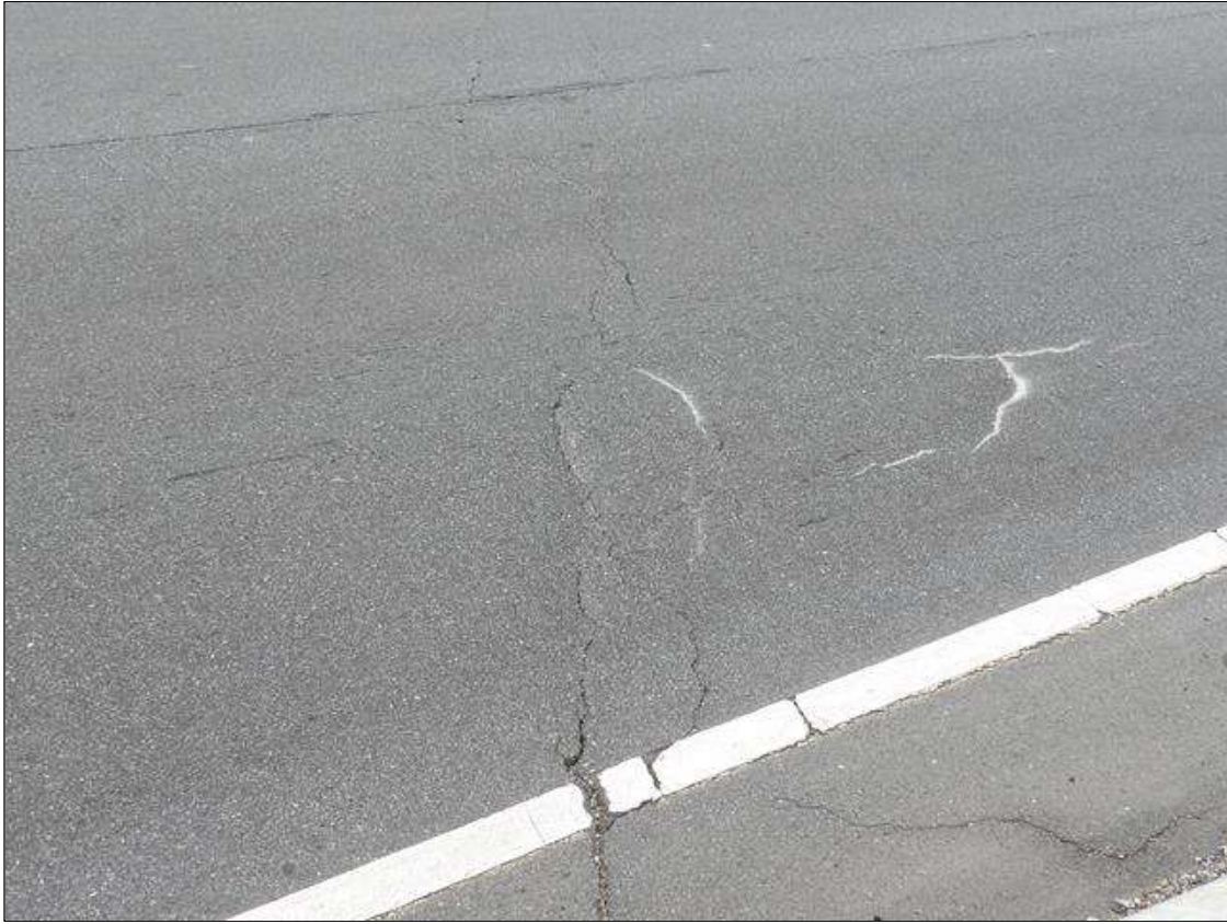
TYPICAL--UP TO 1/8 INCHES TRANSVERSE CRACKS OVER SUBSTRUCTURES END BENT 1 SHOWN
