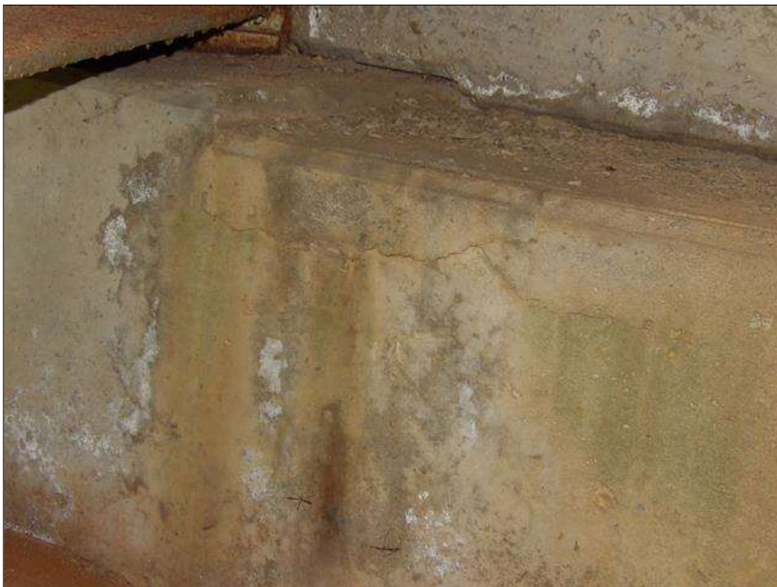
End Bent 1 Cap 1: UP TO 1/16 INCHES HORIZONTAL CRACK IN FACE OF CAP TO LEFT OF BEAM 2
