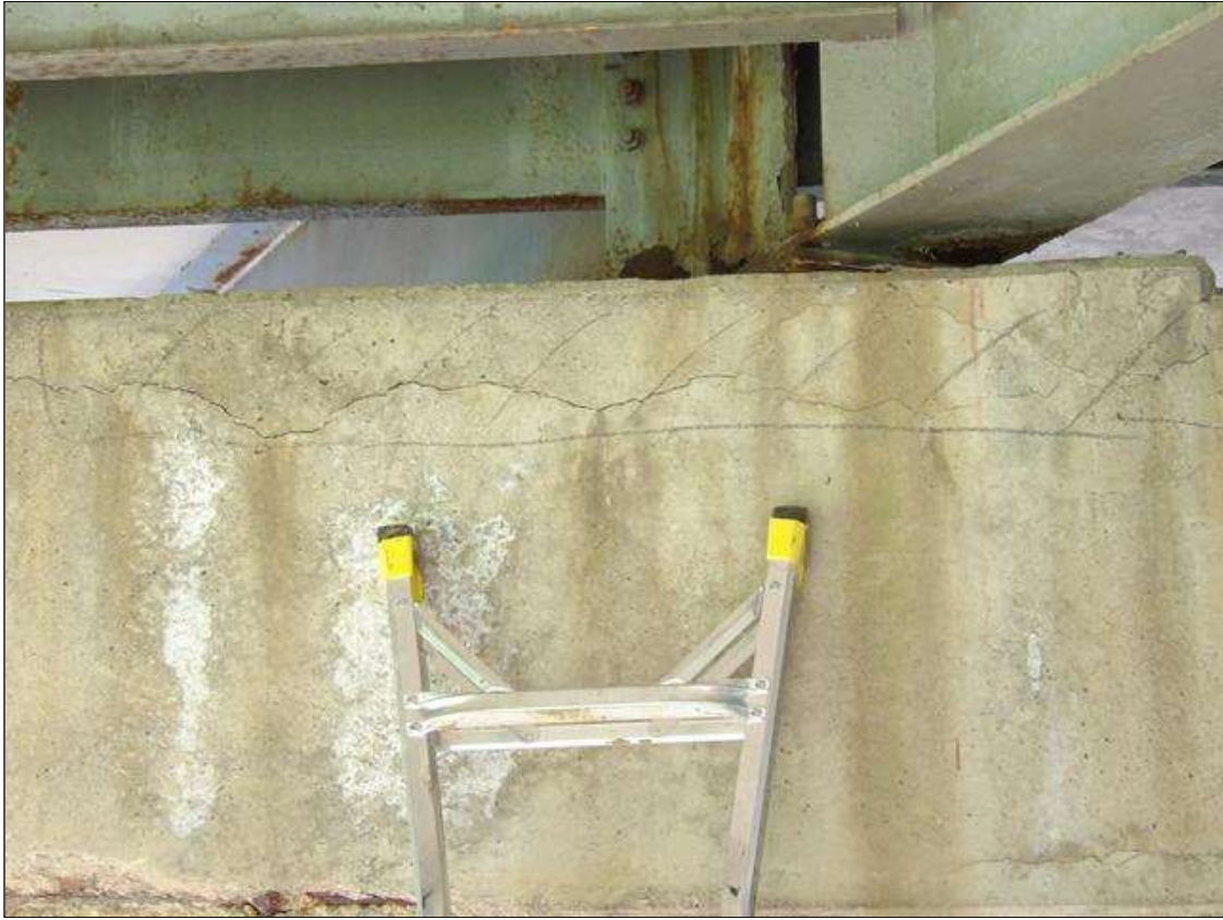
Bent 2 Cap 1: 72 INCHES X 7 INCHES X 11 INCHES AREA OF DELAMINATION WITH UP TO 1/16 INCHES HORIZONTAL CRACKS IN TOP AND SPAN 3 FACE OF CAP BENEATH BEAM 2 AND BAY 2
