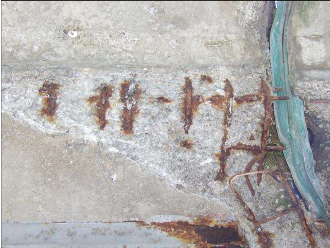
Span 1 Deck: PAR: 53 INCHES X 21 INCHES X 4 INCHES DEEP SPALL WITH EXPOSED REBAR MINOR LOSS IN BOTTOM OF RIGHT OVERHANG ABOVE BENT 1
