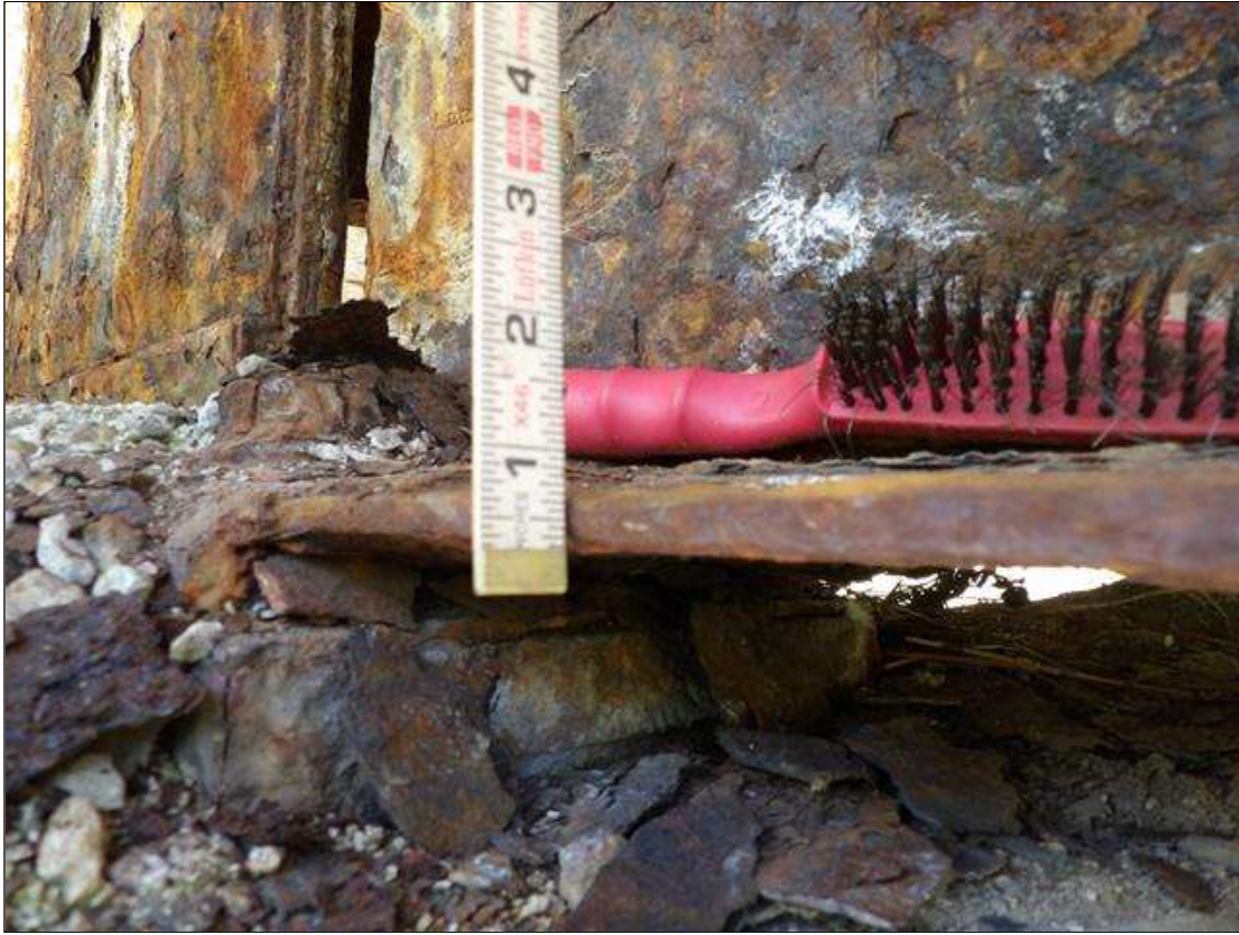
Span 2 Beam 4: PAR: CORROSION ALONG BOTH FACES OF WEB AND BOTTOM FLANGE UP TO 6 FEET LONG X 31 1/2 INCHES HIGH DOWN TO 1/2 INCHES RESIDUAL WEB, AND 6 FEET LONG X 11 1/2 INCHES WIDE DOWN TO 5/16 INCHES RESIDUAL FLANGE AT BENT 1
