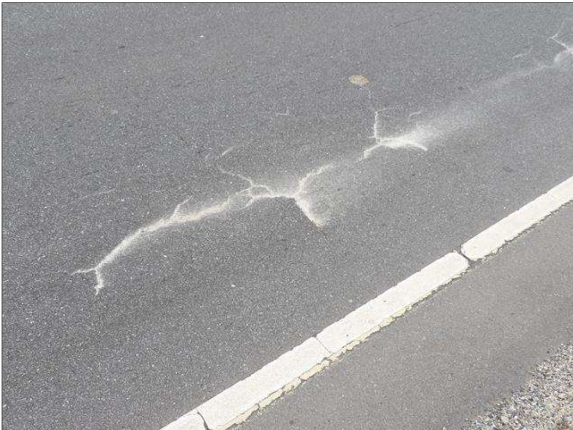
Span 1 Wearing Surface: UP TO 1/32 INCHES TRANSVERSE, LONGITUDINAL AND ALLIGATOR CRACKS IN VARIOUS LOCATIONS
