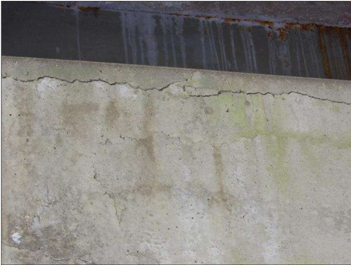
Bent 1 Cap 1: 31 FEET OF UP TO 1/4 INCHES LONGITUDINAL AND HORIZONTAL CRACKS WITH AND WITHOUT EFFLORESCENCE THROUGHOUT TOP, BOTTOM AND SPAN 2 FACE OF CAP
