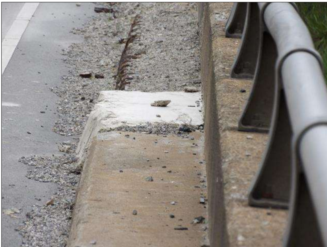
SPAN 2 RIGHT RAIL 3 FOOT X 1 FOOT 5 INCH SOUND PATCH IN CURB AT PIER 1
