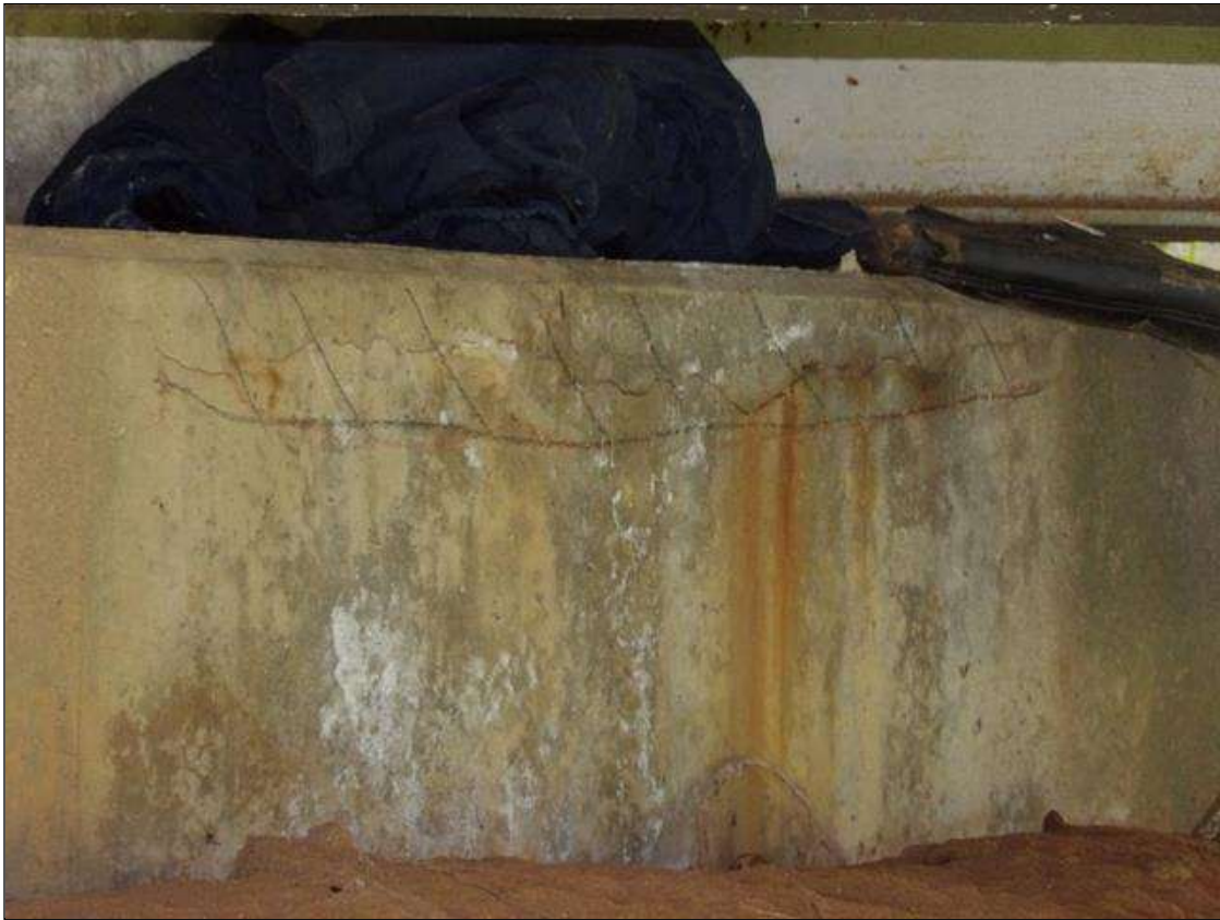
End Bent 1 Cap 1: 55 INCHES X 11 INCHES X 7 INCHES AREA OF DELAMINATION WITH UP TO 1/4 INCHES LONGITUDINAL AND HORIZONTAL CRACKS WITH RUST STAINING IN TOP AND FACE OF CAP BENEATH BAY 1
