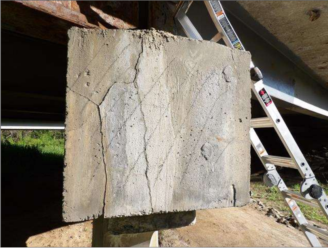
Bent 3 Cap 1: AT RIGHT END, UNSOUND PATCH FULL HEIGHT AND FULL WIDTH WITH CRACKS UP TO 1/8 IN WIDE
