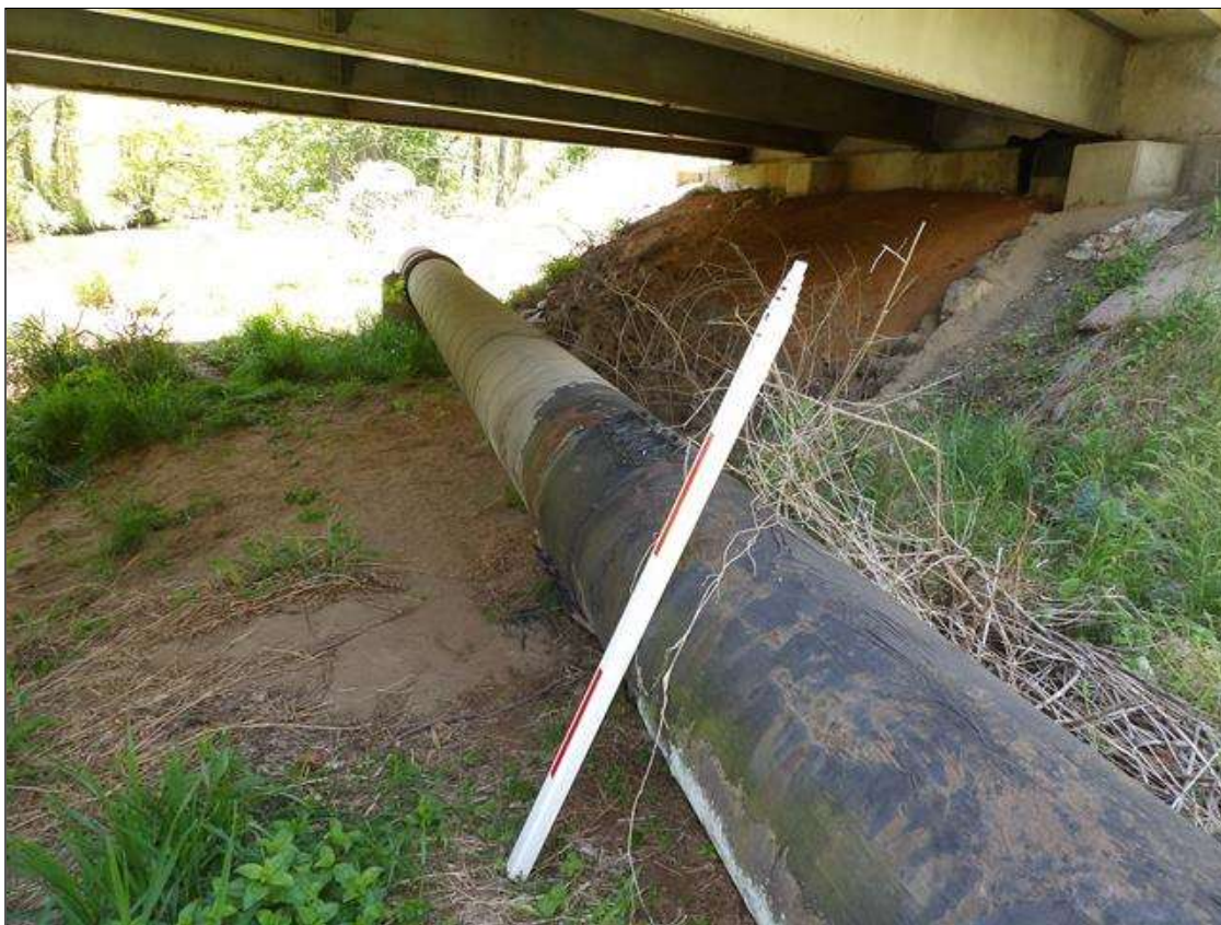
UTILITY UNDER SPAN 1 NOT ATTACHED TO BRIDGE
