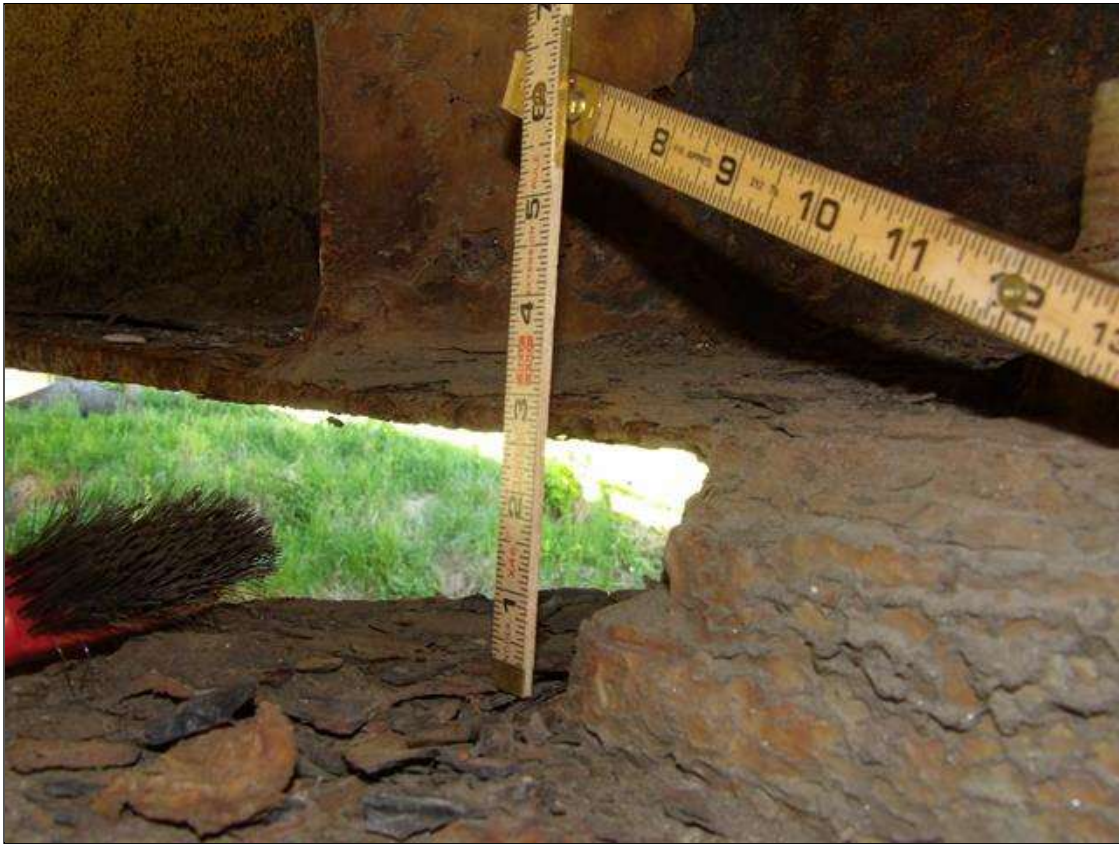
Span 2 Beam 3: PAR: CORROSION ALONG BOTH FACES OF WEB AND BOTTOM FLANGE UP TO 68 INCHES LONG X 7 INCHES HIGH DOWN TO 1/2 INCHES RESIDUAL WEB, AND 60 INCHES LONG X 11 1/2 INCHES WIDE DOWN TO 3/16 INCHES RESIDUAL FLANGE AT BENT 2
