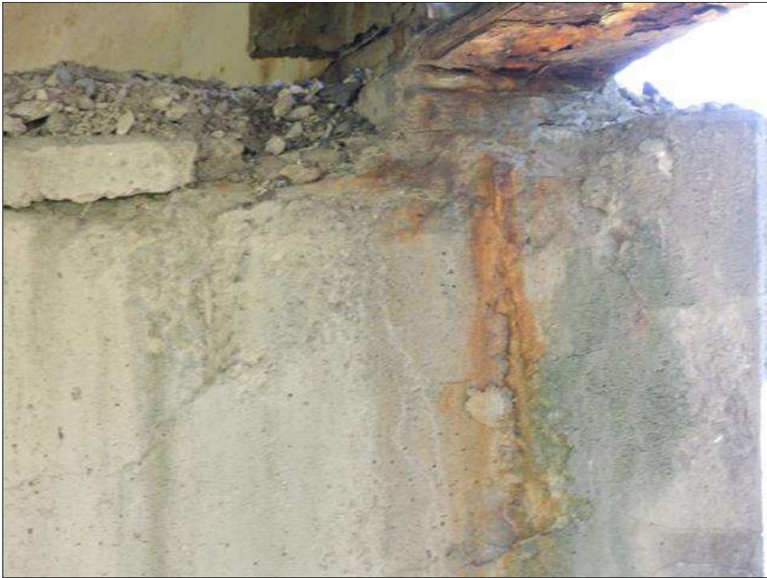
Bent 2 Cap 1: PAR: 48 INCHES X 22 INCHES X 3 INCHES DEEP SPALL WITH EXPOSED REBAR IN SPAN 2 FACE OF CAP BENEATH BEAM 4 WITH 5 PERCENT BEARING LOSS
