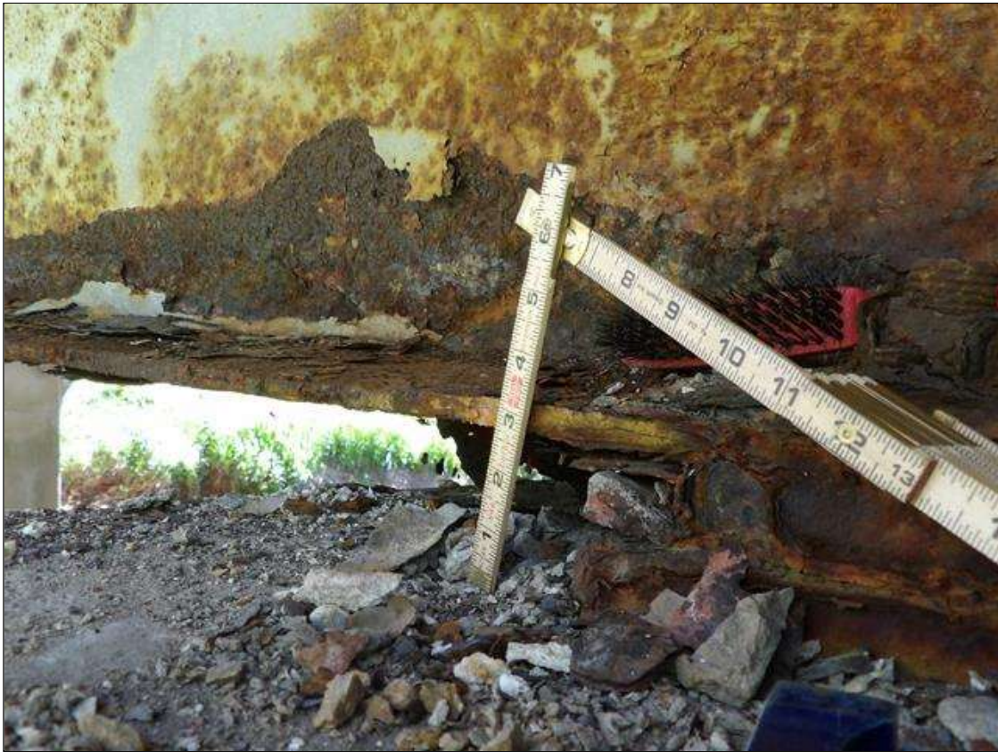
Span 2 Beam 1: PAR: CORROSION ALONG BOTH FACES OF WEB AND BOTTOM FLANGE UP TO 36 INCHES LONG X 6 INCHES HIGH DOWN TO 1/2 INCHES RESIDUAL WEB, AND 36 INCHES LONG X 11 1/2 INCHES WIDE DOWN TO 7/16 INCHES RESIDUAL FLANGE AT BENT 1
