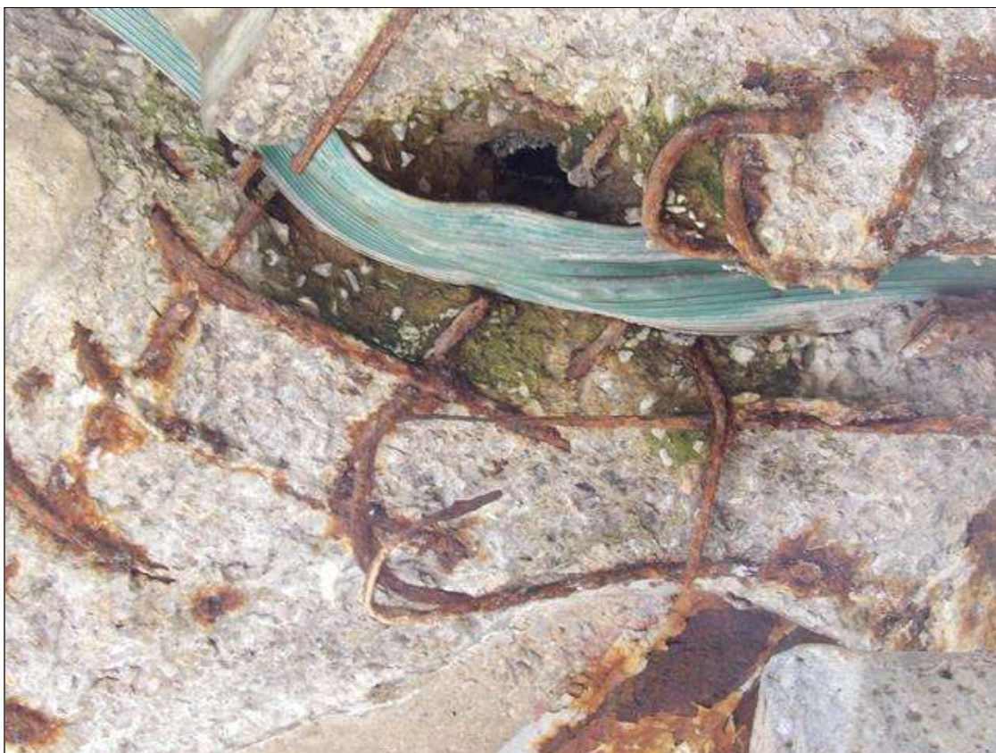
PAR--SPAN 1 BENT 1 RIGHT OVERHANG DIAPHRAGM, SPALL 1 FEET LONG X 2 FEET WIDE X FULL DEPTH WITH EXPOSED REBAR WITH 70 PERCENT SECTION LOSS
