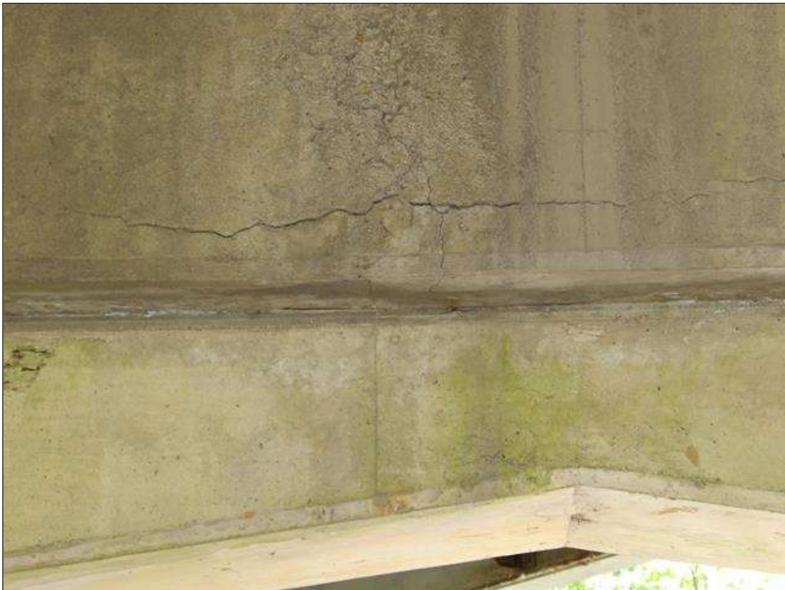
Bent 1 Cap 1: 41 INCHES X 6 INCHES X 14 INCHES AREA OF DELAMINATION WITH UP TO 1/16 INCHES HORIZONTAL AND VERTICAL CRACKS IN BOTTOM AND SPAN 1 FACE OF CAP AT MID LENGTH
