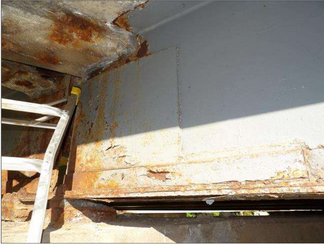
TYPICAL BEAM 4-- WELDED PLATE REPAIR AT BENT 3 BOTTOM FLANGE HAS A 3 FOOT 3 INCH X 4 INCH X 4 INCH X 1/2 INCH ANGLE ON RIGHT AND 2 FOOT X 4 INCH X 4 INCH X 1/2 INCH ON LEFT AND WEB HAS A 24 INCH X 24 INCH X 1/2 INCH ON RIGHT SIDE, SPAN 1 FAR, SPAN 2 FAR, SPAN 3 AND SPAN 4 NEAR
