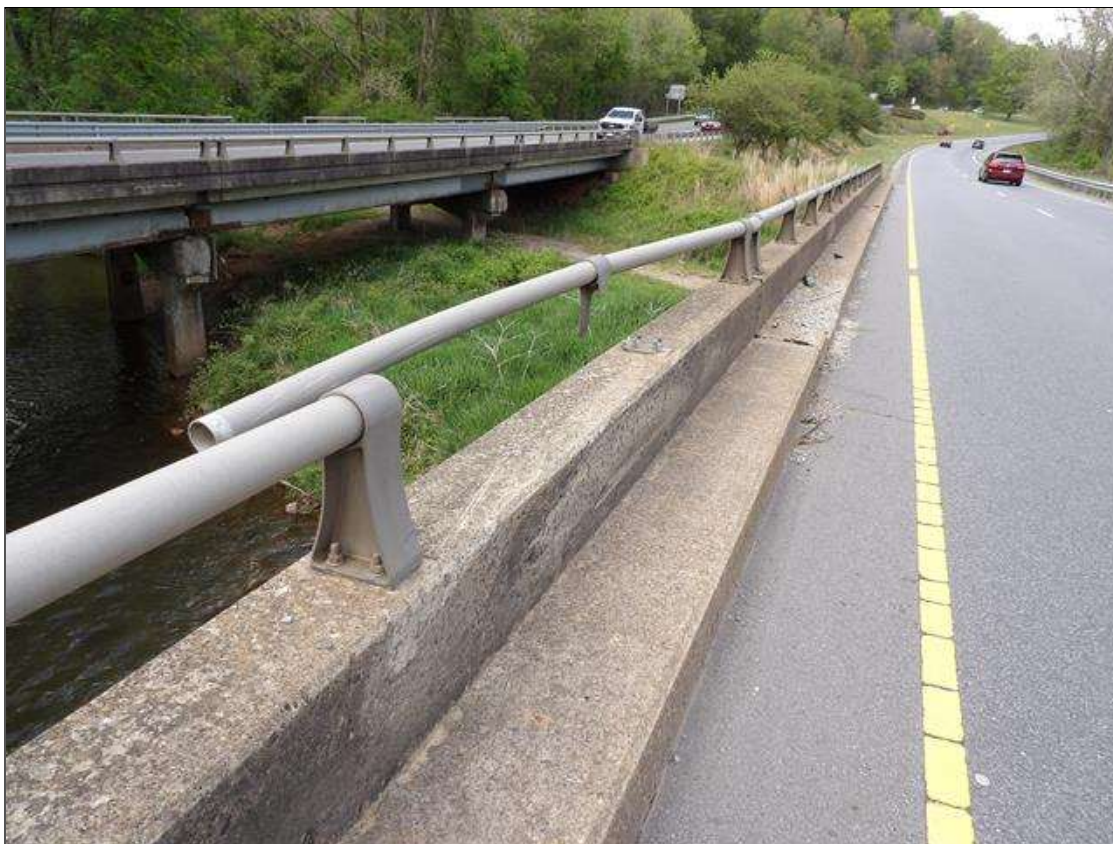
Span 2 Left Bridge Rail: PAR--IMPACT DAMAGE TO RAIL AND POST AT PIER 2, RAIL IS BROKEN/SEPARATED AND RAIL POSTS IS DISCONNECTED FROM BRIDGE
