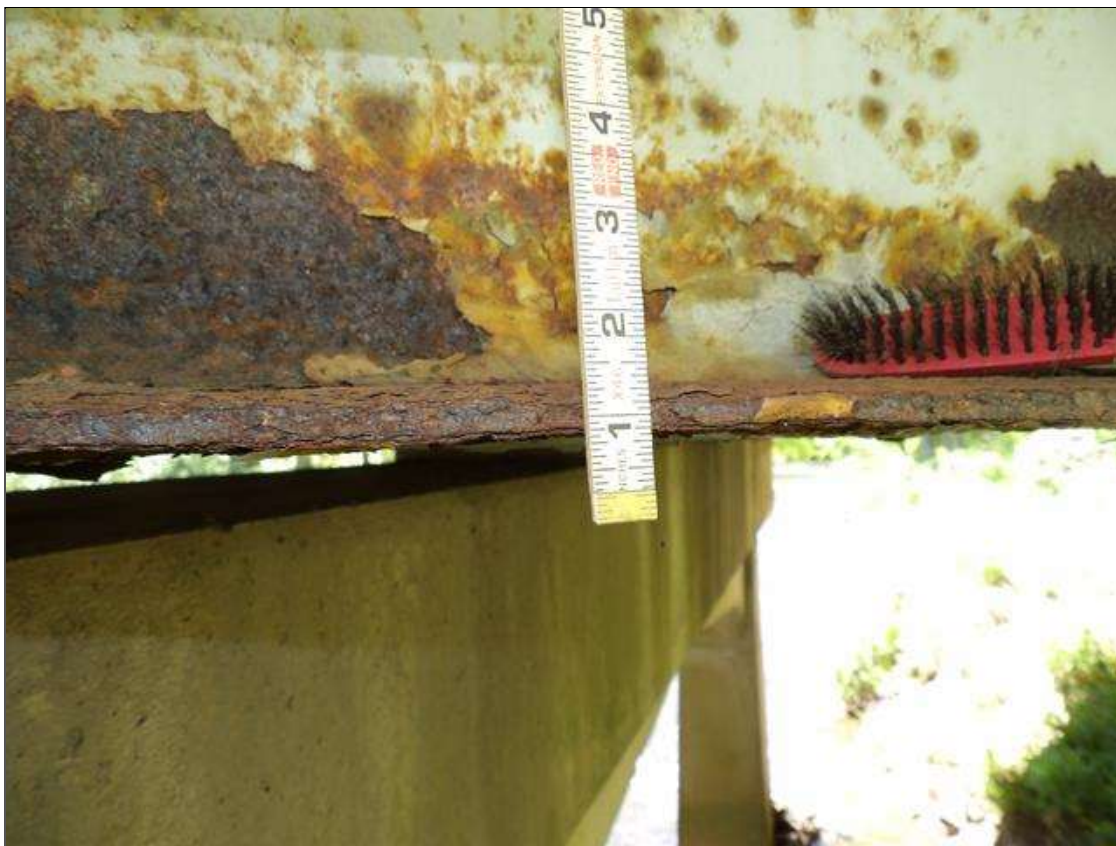
Span 1 Beam 1: PAR: CORROSION ALONG BOTH FACES OF WEB AND BOTTOM FLANGE UP TO 29 INCHES LONG X 10 INCHES HIGH DOWN TO 1/2 INCHES RESIDUAL WEB, AND 30 INCHES LONG X 11 1/2 INCHES WIDE DOWN TO 3/8 INCHES RESIDUAL FLANGE AT BENT 1
