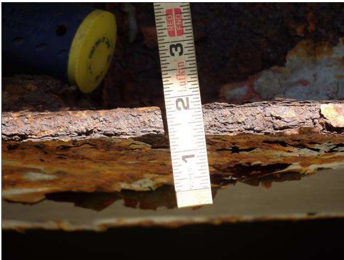
Span 3 Beam 4: PAR--CORROSION ALONG RIGHT FACE OF WEB AND BOTTOM FLANGE UP TO 24 INCHES LONG X 4 INCHES HIGH DOWN TO 1/2 INCHES RESIDUAL WEB, AND 24 INCHES LONG X 5 1/2 INCHES WIDE DOWN TO 3/8 INCHES RESIDUAL FLANGE, EXTENDING FROM PLATE REPAIR 4 FEET FROM BENT 2
