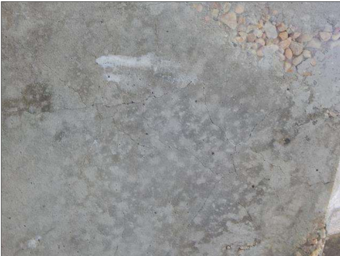
Span 1 Deck: 12' x 2' area of hairline longitudinal and transverse cracks in North overhang (South overhang similar)
