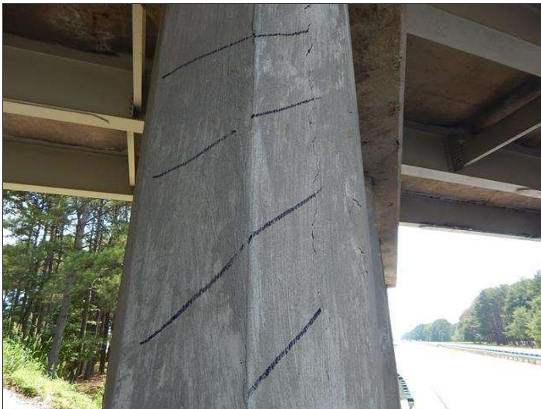
Bent 3 Pile 2: 4' x 1' area of delamination with 7' up to 1/16" vertical crack on North face
