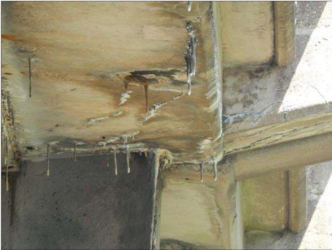
Span 3 Deck: 6' hairline longitudinal and diagonal cracks with efflorescence in South overhang at Bent 3
