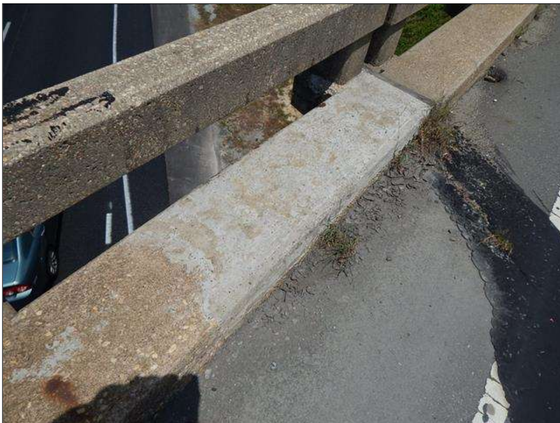
Span 3 Left Bridge Rail: 7' x 2' area of repaired section of curb at Bent 3
