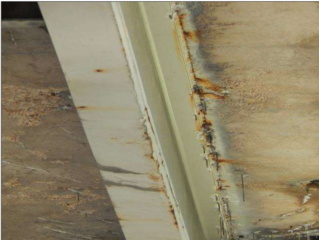
Span 3 Beam 4: 25' surface rust on both flanges
