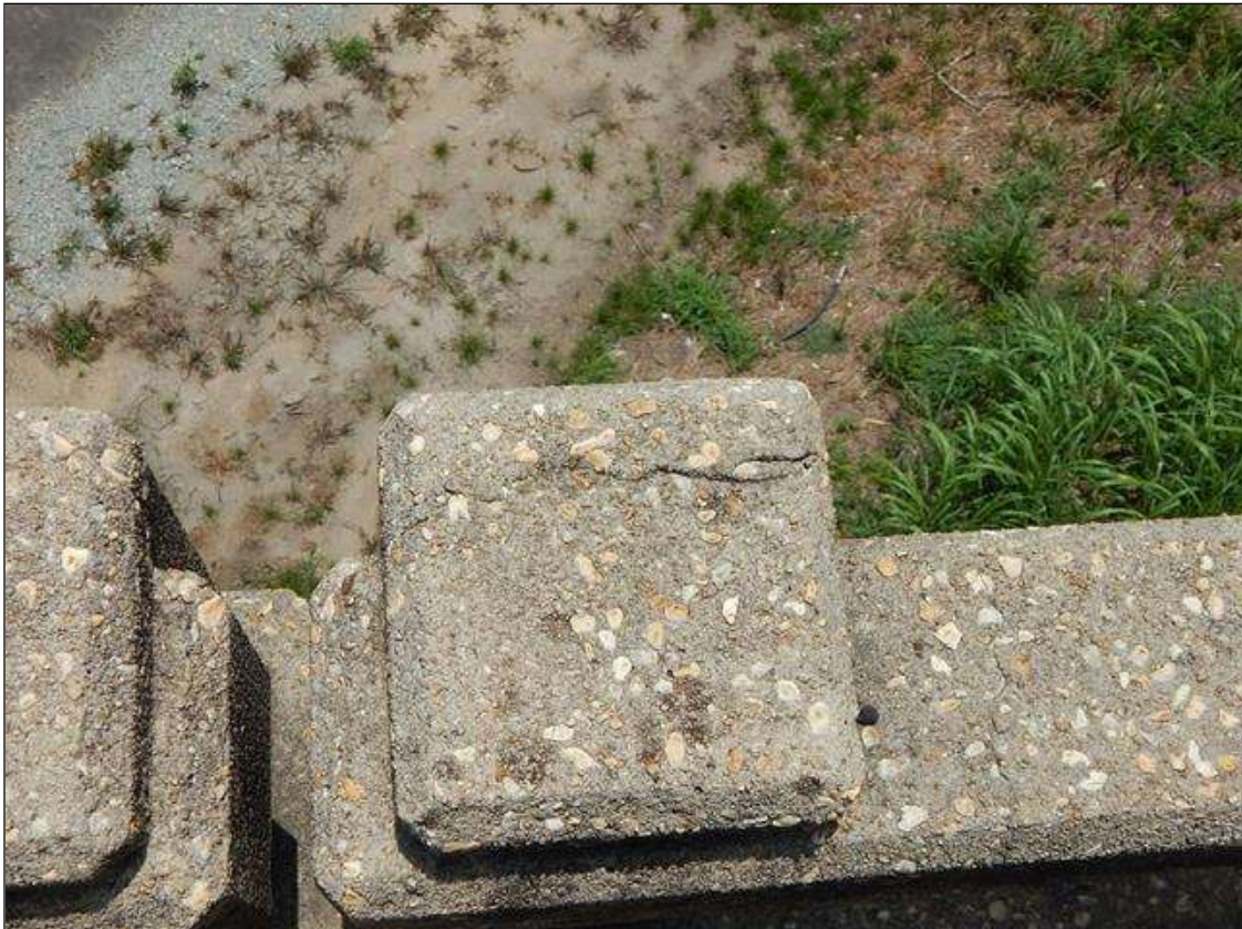
Span 1 Right Bridge Rail: 10" up to 1/8" longitudinal crack on top of Post 5
