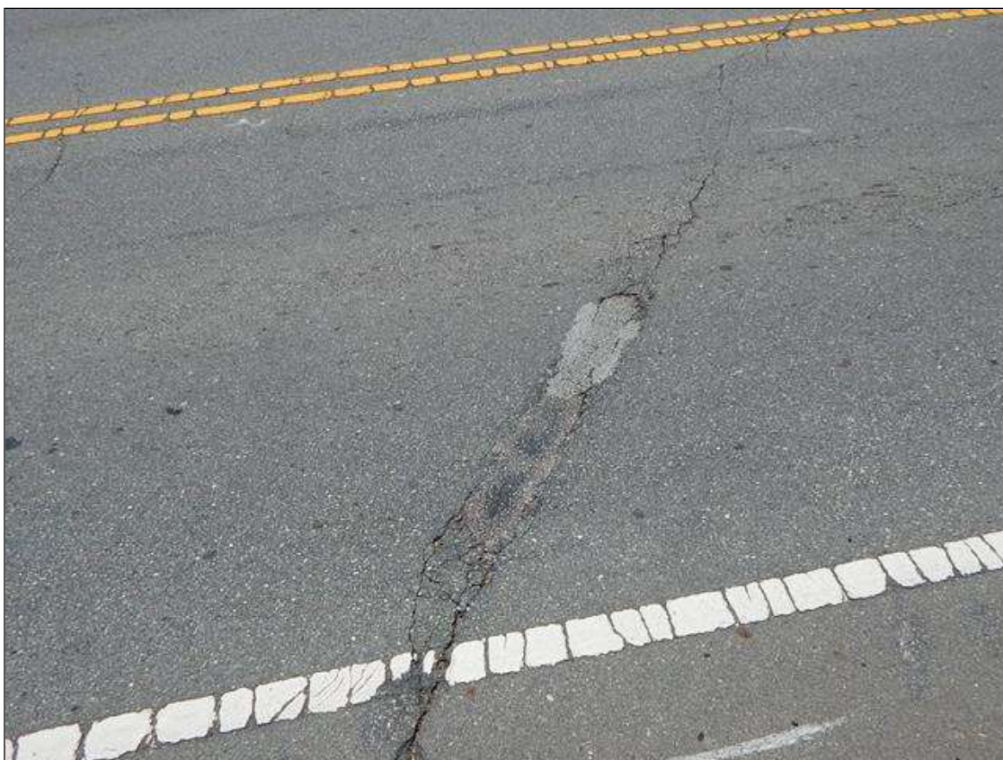
Span 1 Wearing Surface: 8" x 50" area of patch with 1/16" transverse cracks in Eastbound lane at End Bent 1
