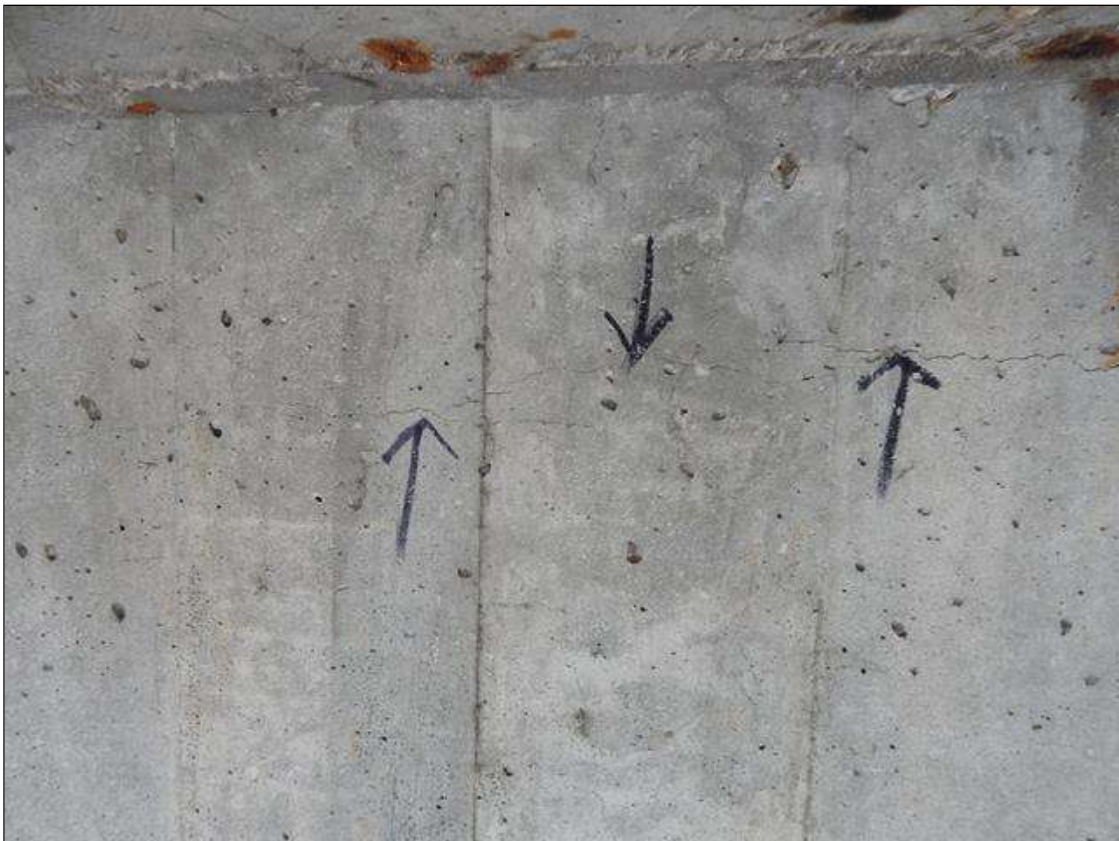
End Bent 1 Abutment/Backwall : 5' hairline horizontal crack in Bay 1
