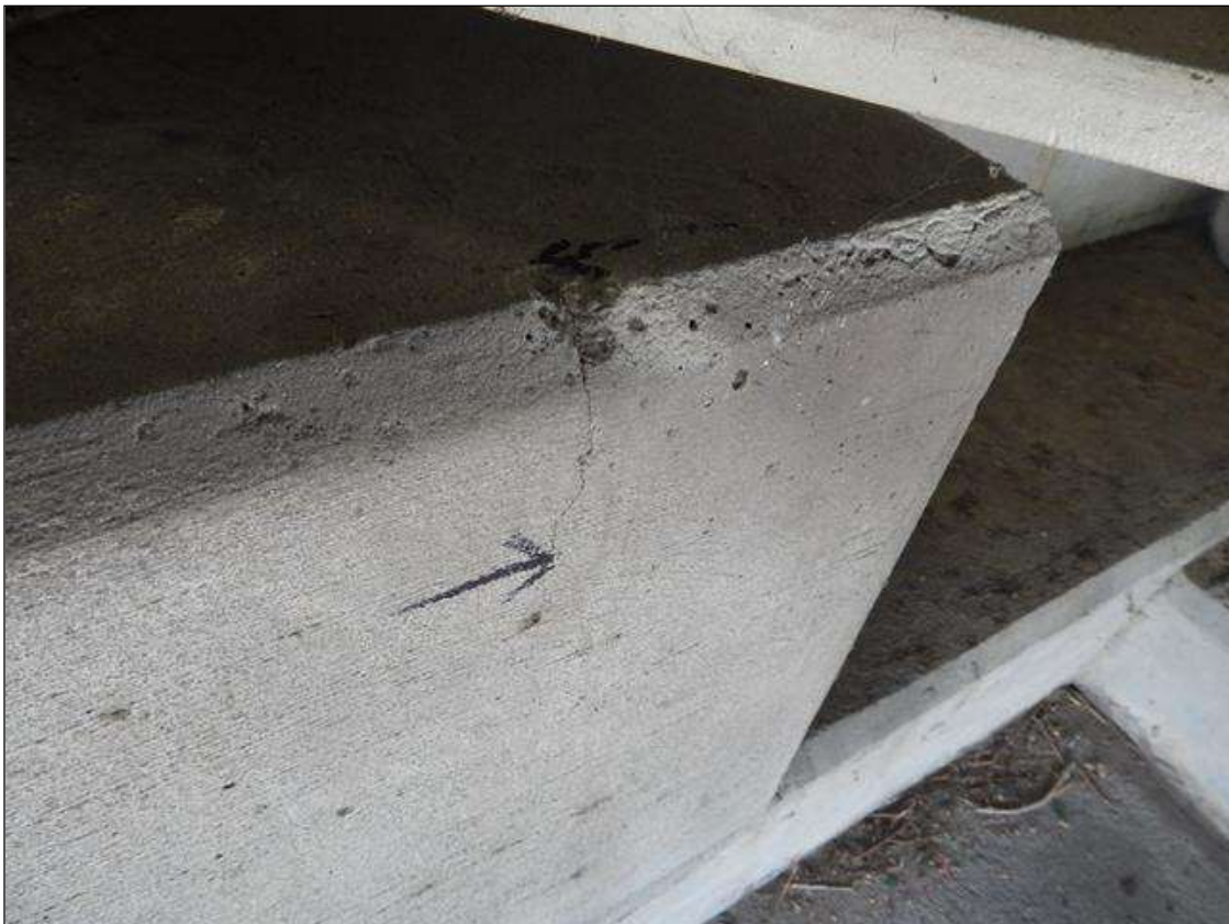
End Bent 2 Cap 1: 22" hairline vertical and longitudinal crack on Beam 2 pedestal
