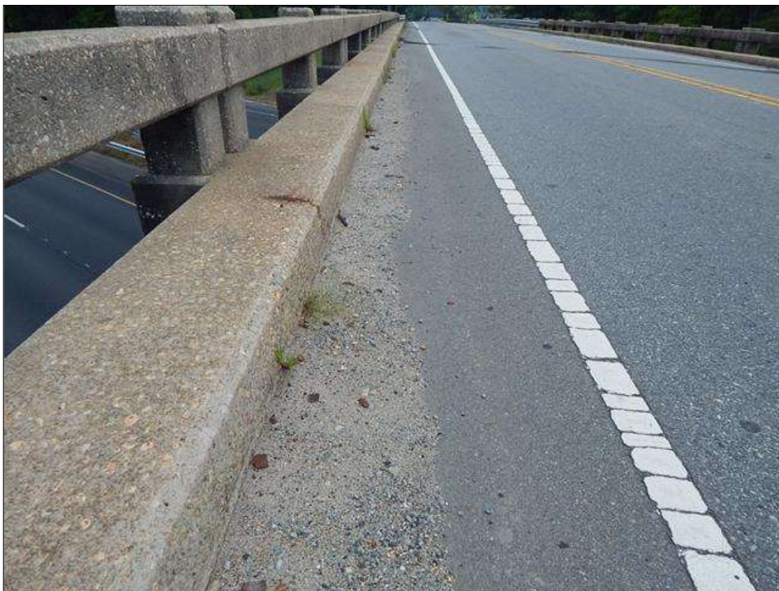
Full length x 15" dirt and debris in North gutter (South gutter similar)
