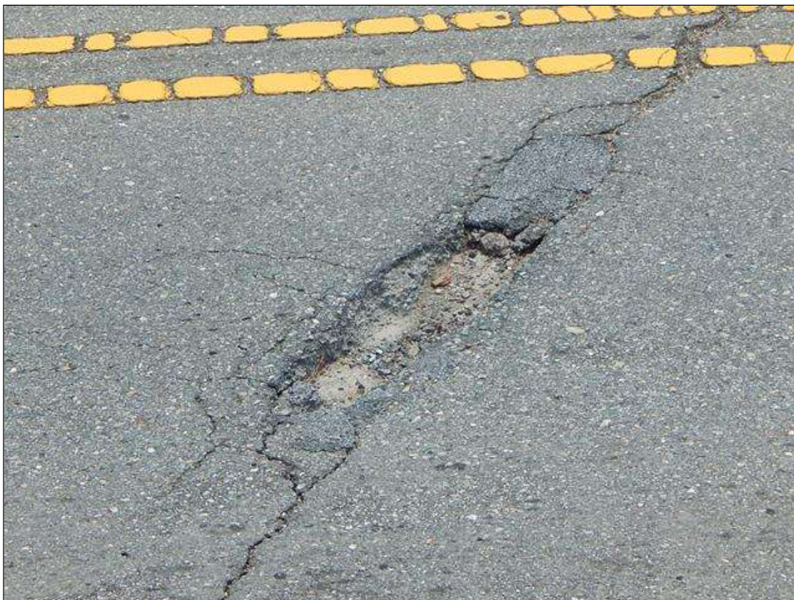
Span 4 Wearing Surface: (2) up to 29" x 8" x 3" deep area of missing asphalt wearing surface at End Bent 2
