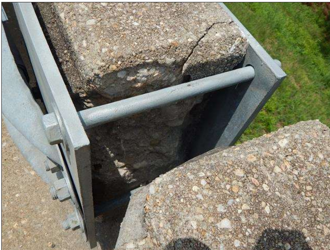
Span 1 Right Bridge Rail: 3" x 16" x 11" deep spall in rail and Post 2
