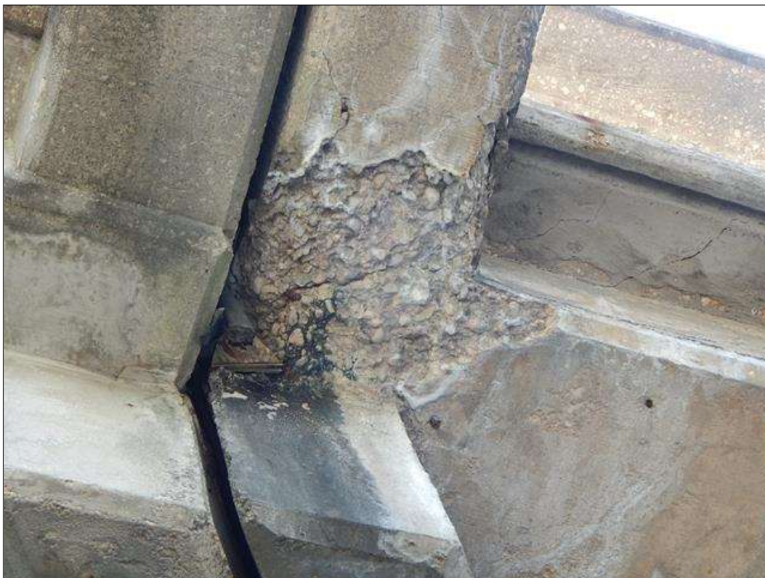
Span 3 Deck: 16" x 20" x 1 1/2" deep spall on North overhang at Bent 3
