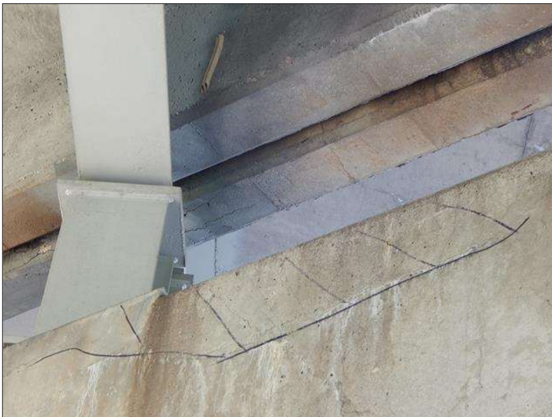
Bent 3 Cap 1: 7' x 1' area of delamination on Span 4 face under Bay 1 (Span 3 face similar)
