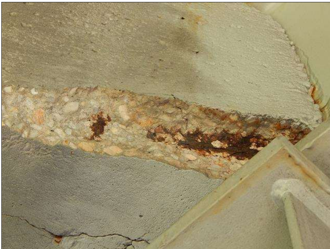
Span 4 Beam 3: 18" x 5" x 2" deep spall with exposed rebar on Bent 3 diaphragm in Bay 3
