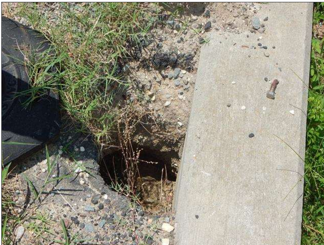
(2) up to 20" x 9" x 20" deep erosion behind Northwest wingwall
