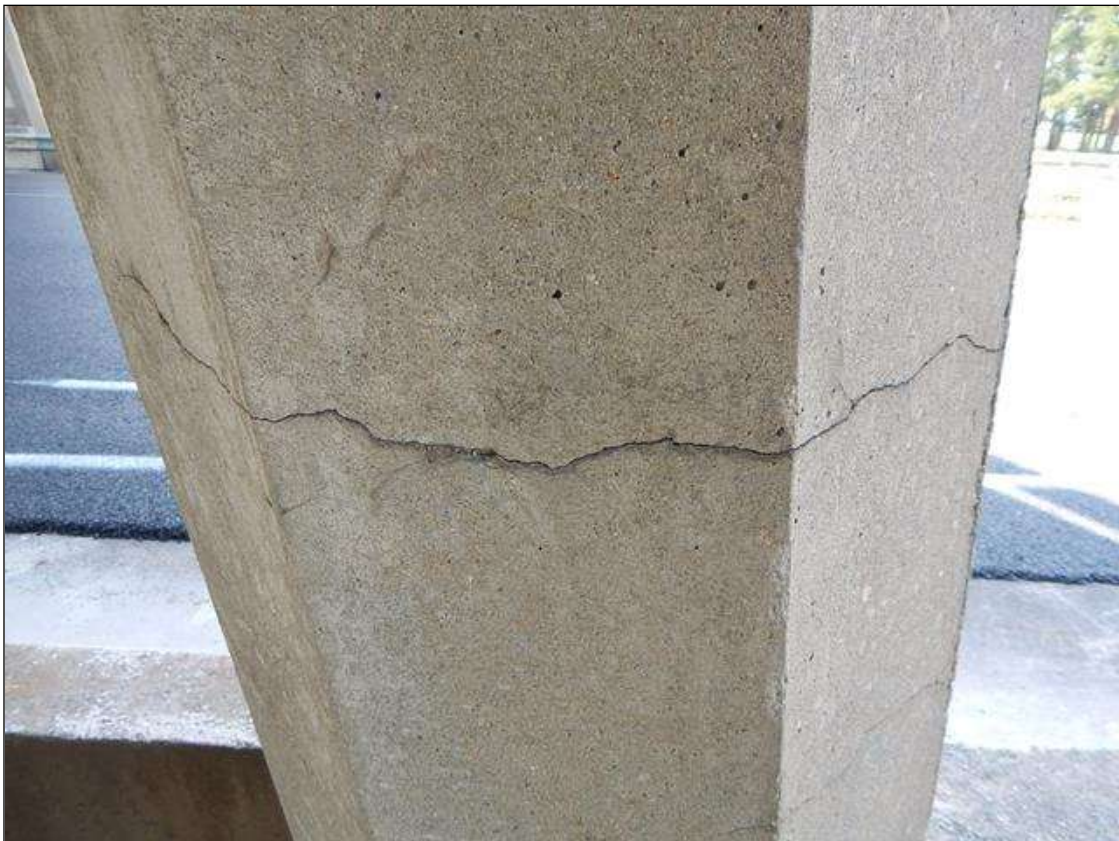
Bent 3 Pile 1: (3) up to 35" hairline horizontal cracks on Span 4 face
