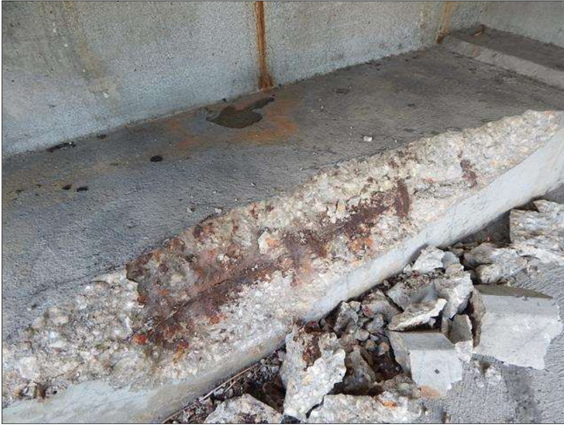
End Bent 2 Cap 1: 67" x 12" x 7" deep spall with exposed rebar under Bay 1 (PM)
