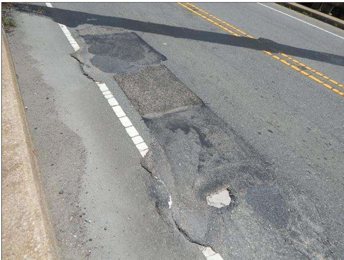
Span 3 Wearing Surface: 15' x 4' area of patch with (2) up to 8" x 12" x 2" deep spalls in Eastbound lane at Bent 3
