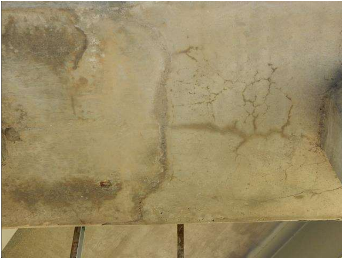
Bent 3 Cap 1: 34' x up to 3' area of hairline longitudinal and transverse cracks on bottom of cap
