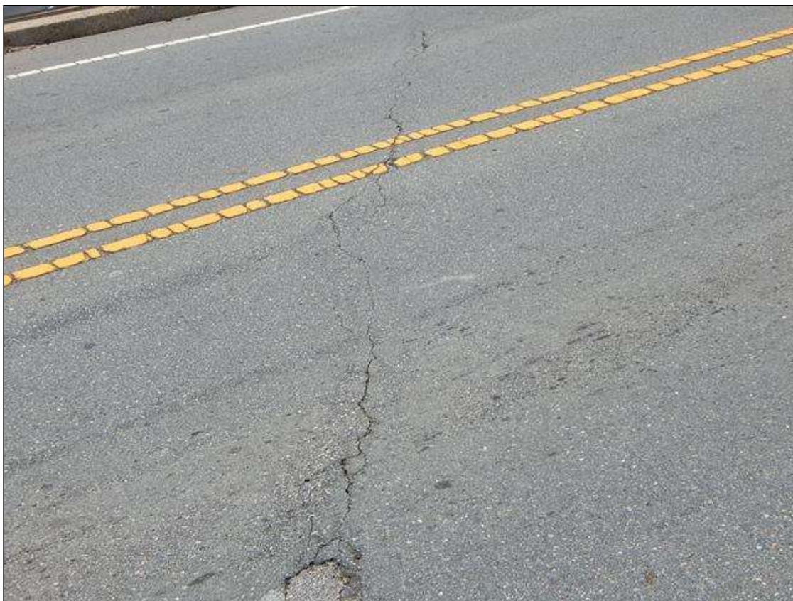
Span 1 Wearing Surface: 34 square feet up to 1/16" transverse cracks at End Bent 1
