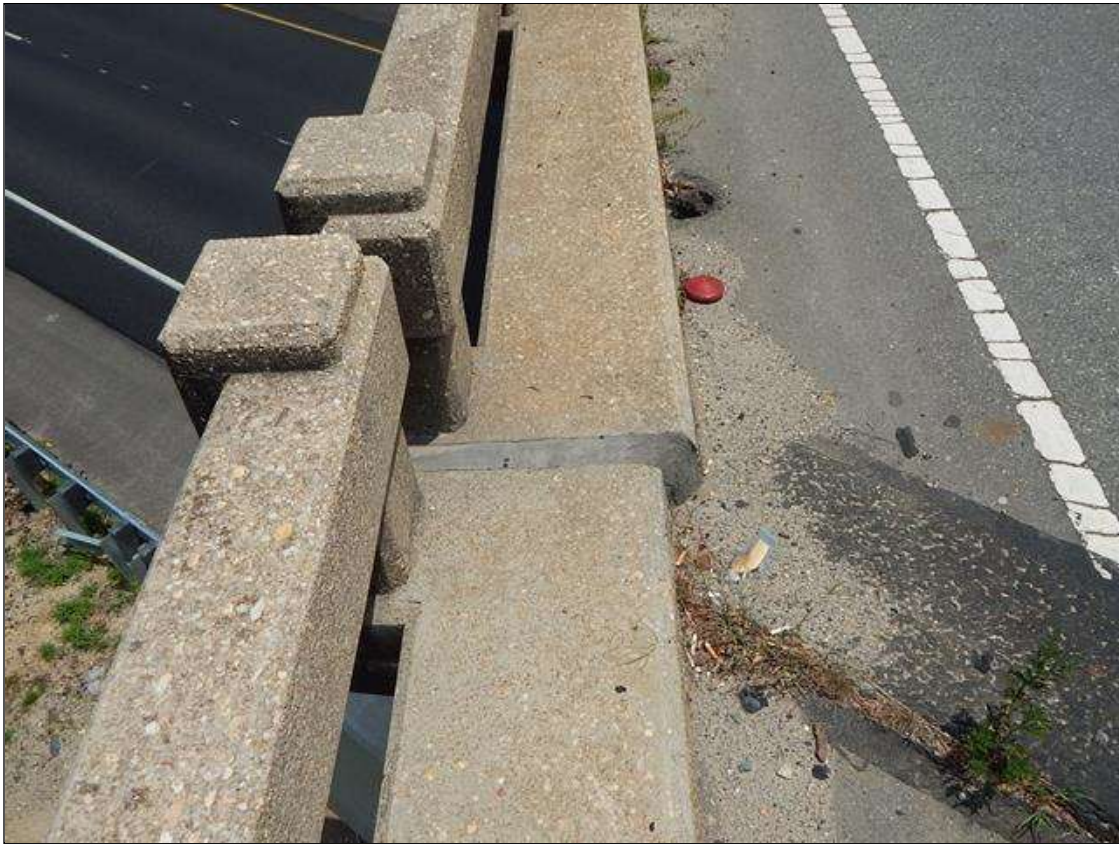
Span 1 Left Bridge Rail: 3" rotation to the North
