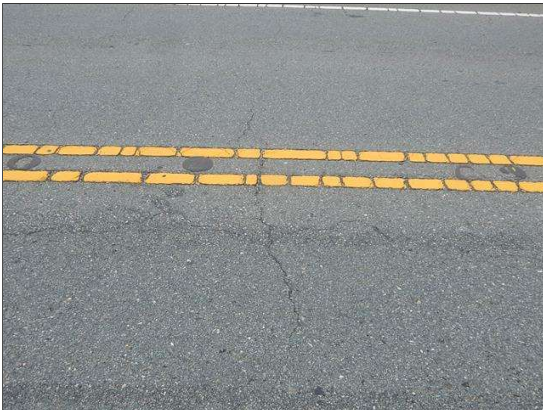
Span 1 Wearing Surface: 90 square feet up to 1/16" longitudinal and transverse cracks
