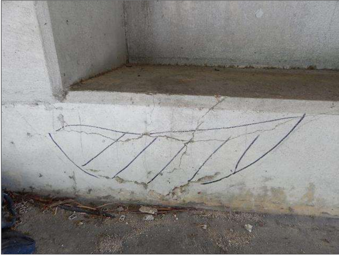
End Bent 2 Cap 1: 28" x 10" area of delamination under Bay 3
