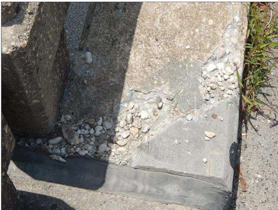
Span 3 Right Bridge Rail: 20" x 22" x 1" deep spall on curb at Bent 3
