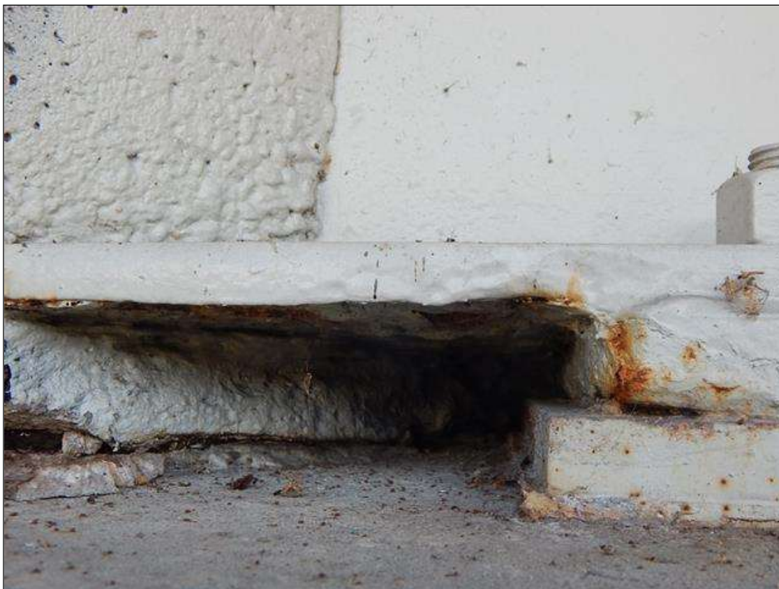
Span 4 Beam 1: 8" x 8" area of 1/4" section loss (11/16" remaining) on left side of bottom flange at End Bent 2 (PM)
