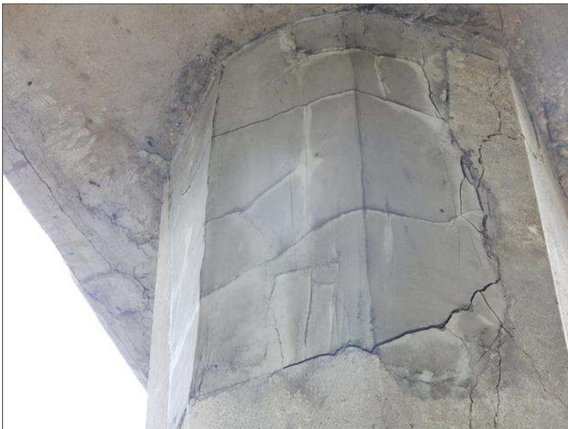
Bent 2 Pile 6: 2' x 2' area of patch with 1/8" vertical and horizontal cracks on North face
