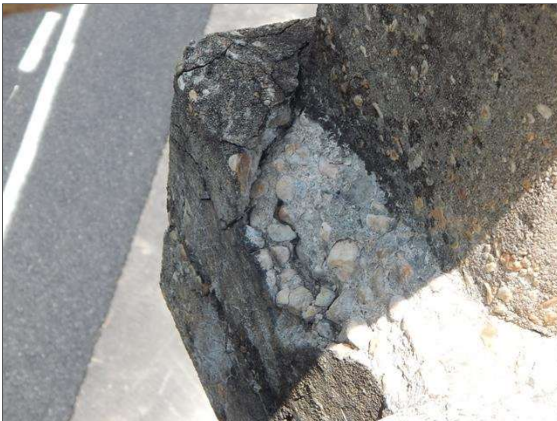
Span 3 Left Bridge Rail: 3" x 10" x 4" deep spall on Post 12 connection bracket
