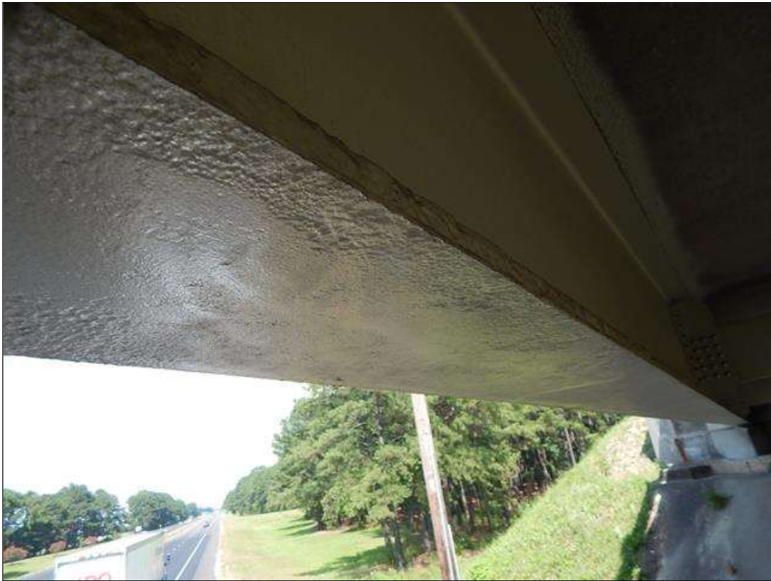
Span 4 Beam 1: 42" up to 1/16" pitting with no rust on bottom flange at Bent 3
