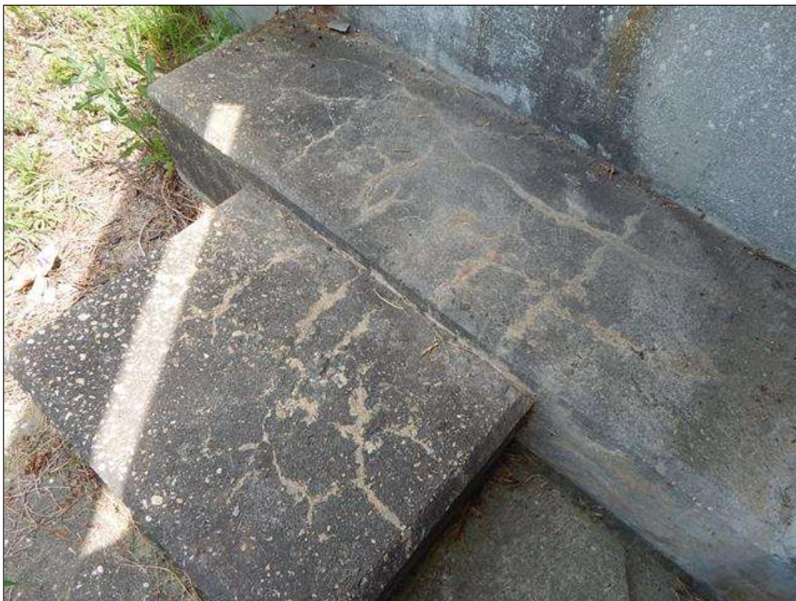
End Bent 2 Cap 1: 5' x 4' area of hairline longitudinal and transverse cracks on top of cap at North end
