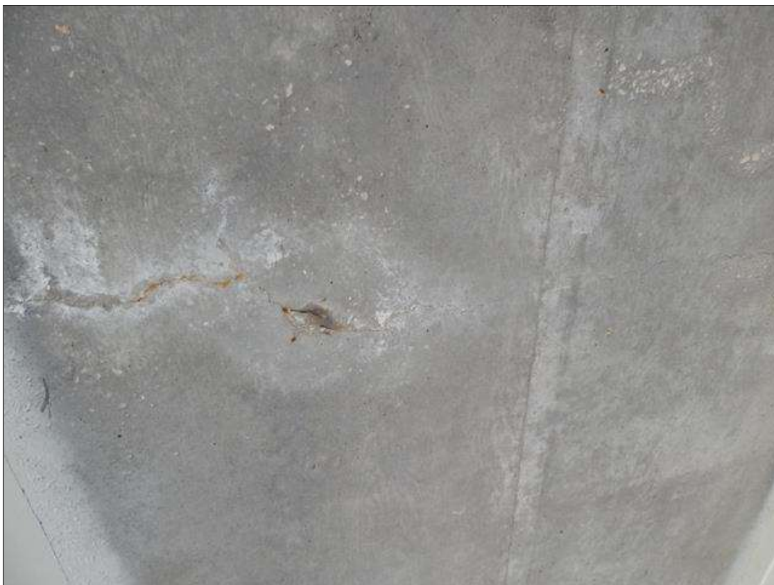
Span 4 Deck: 56 square feet hairline transverse cracks with efflorescence in bottom of deck
