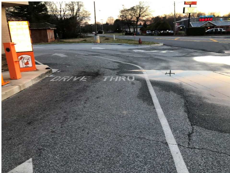
Photo 4: Looking southeast showing asphalt cracking.
