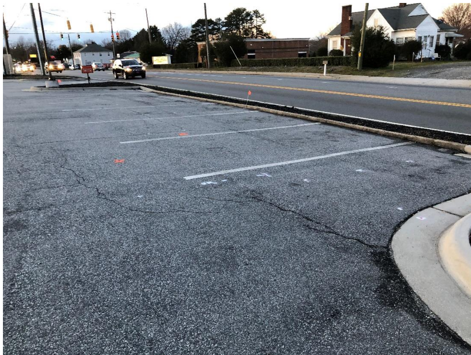
Photo 14: Looking north at parking area along Old Hollow Rd. showing GPR anomaly and unknown utility near proposed boring locations.
