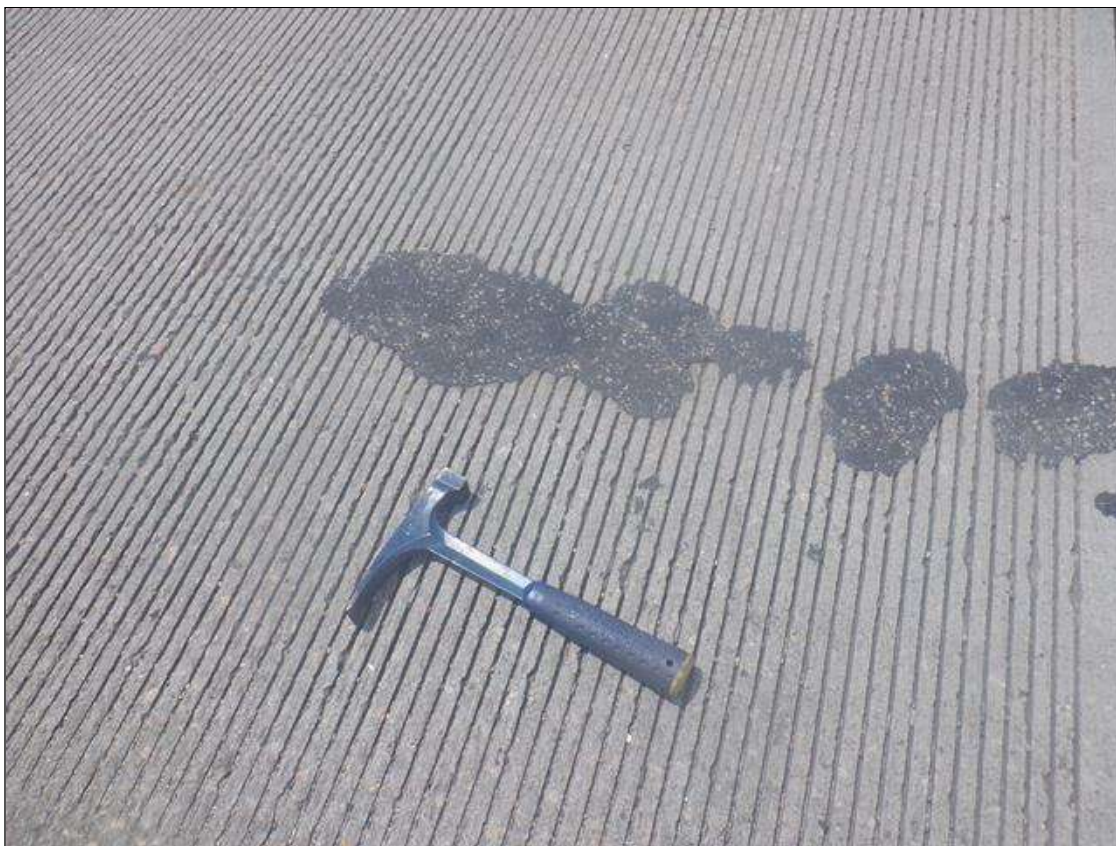
Span 2 Deck: UP TO 20 SQ FT OF ASPHALT PATCHED AREAS IN SCATTERED LOCATIONS.
