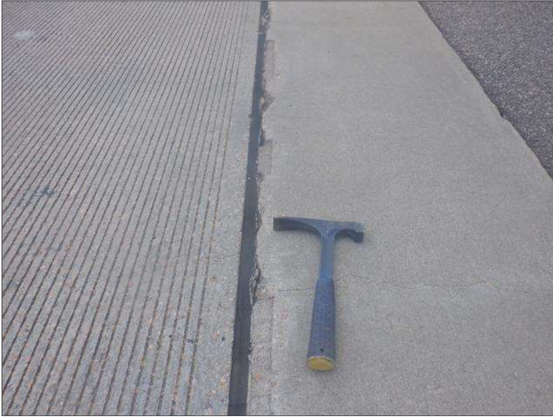
Span 4 Expansion Joint: SCATTERED ALONG THE LENGTH, EDGE CHIPPING UP TO 3/4" WIDE X 3/4" DEEP WITH LOSS OF SEAL ADHESION [LOSS OF SEAL ADHESION IS ALSO PRESENT IN SCATTERED AREAS OF EDGE PATCHING]
