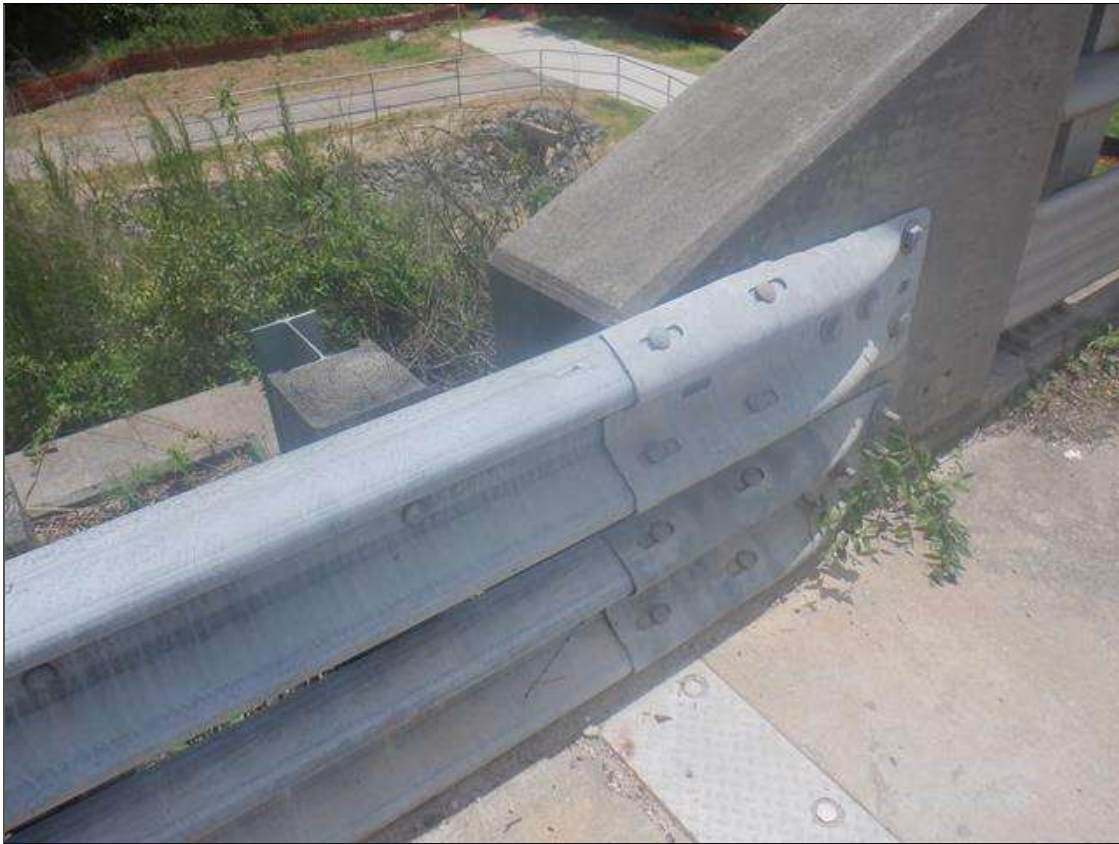
GUARDRAIL TO BRIDGE RAIL CONNECTION AT NORTHEAST CORNER SIMILAR AT SOUTHEAST CORNER
