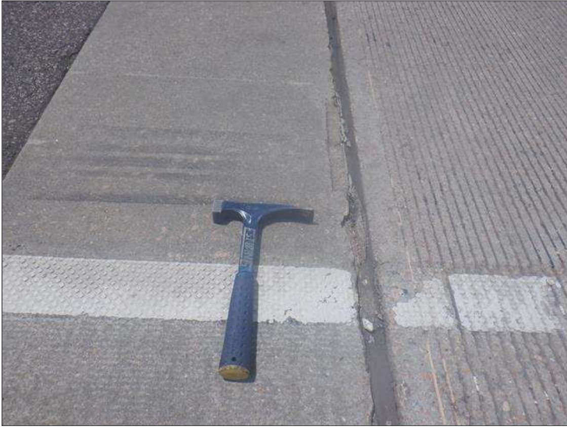
Span 1 Expansion Joint: SCATTERED ALONG THE LENGTH, EDGE CHIPPING UP TO 3/4" WIDE X 3/4" DEEP WITH LOSS OF SEAL ADHESION [LOSS OF SEAL ADHESION IS ALSO PRESENT IN SCATTERED AREAS OF EDGE PATCHING]
