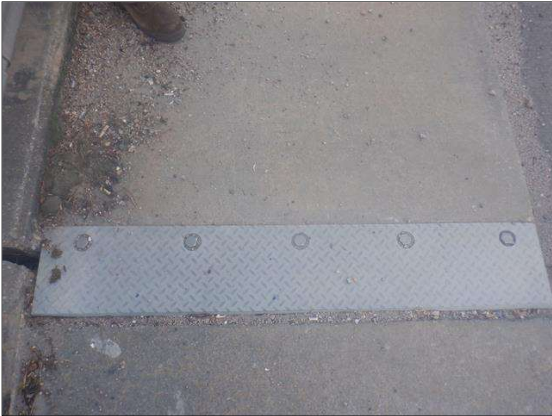
STEEL PLATE IN SIDEWALK AT BENT 2
