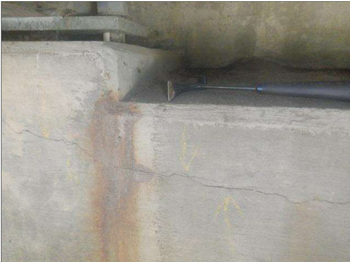
End Bent 2 Cap 1: 3' X UP TO 1/32" LONGITUDINAL CRACK, SOUTH FACE, BENEATH BEAM 3.
