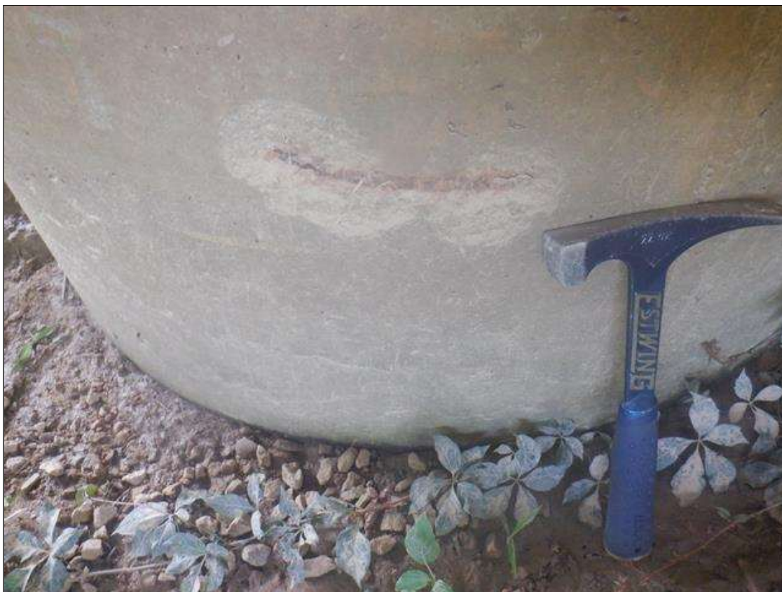
Bent 3 Pile 2: 8 IN LONG X UP TO 4 IN WIDE X 1/2 IN DEEP SPALL, WITH EXPOSED REINFORCING, EAST FACE, 8' FROM BOTTOM OF CAP [NO MEASURABLE SECTION LOSS]
