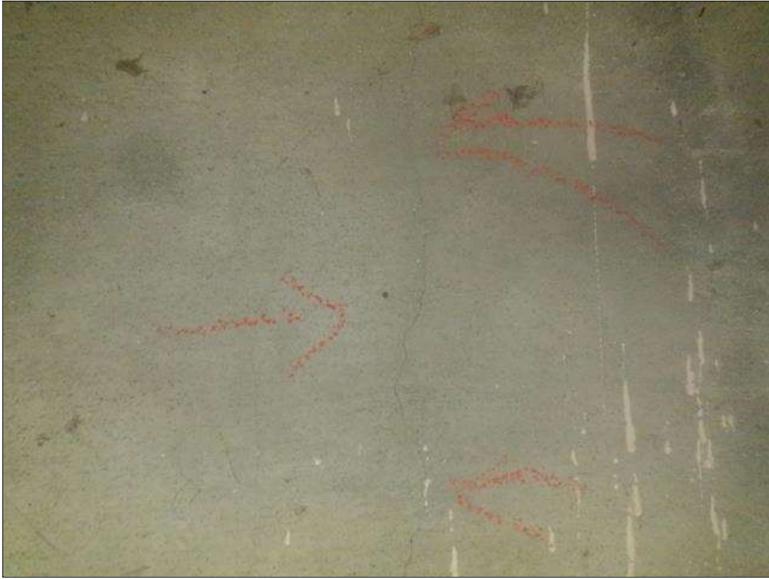
End Bent 1 Abutment: TWO (2) FULL HEIGHT X 1/64 IN WIDE VERTICAL CRACKS IN THE BACKWALL AT RANDOM.
