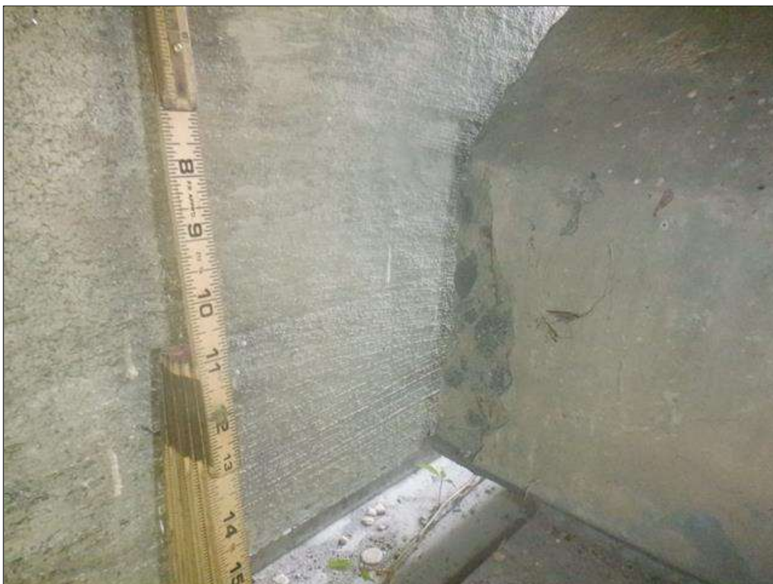
Span 1 Beam 1: RIGHT BOTTOM FLANGE AT ABUTMENT 1, SPALL APPROXIMATELY 2 IN LONG X 8 IN HIGH X UP TO 1/2 DEEP
