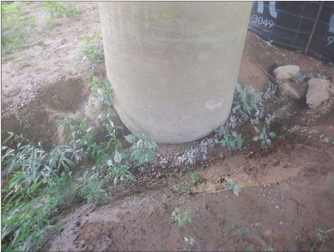
SOIL EROSION AROUND BENT 3 PILE 2 UP TO 7 FT IN DIAMETER X 2 FT DEEP DUE TO SCOUR.
