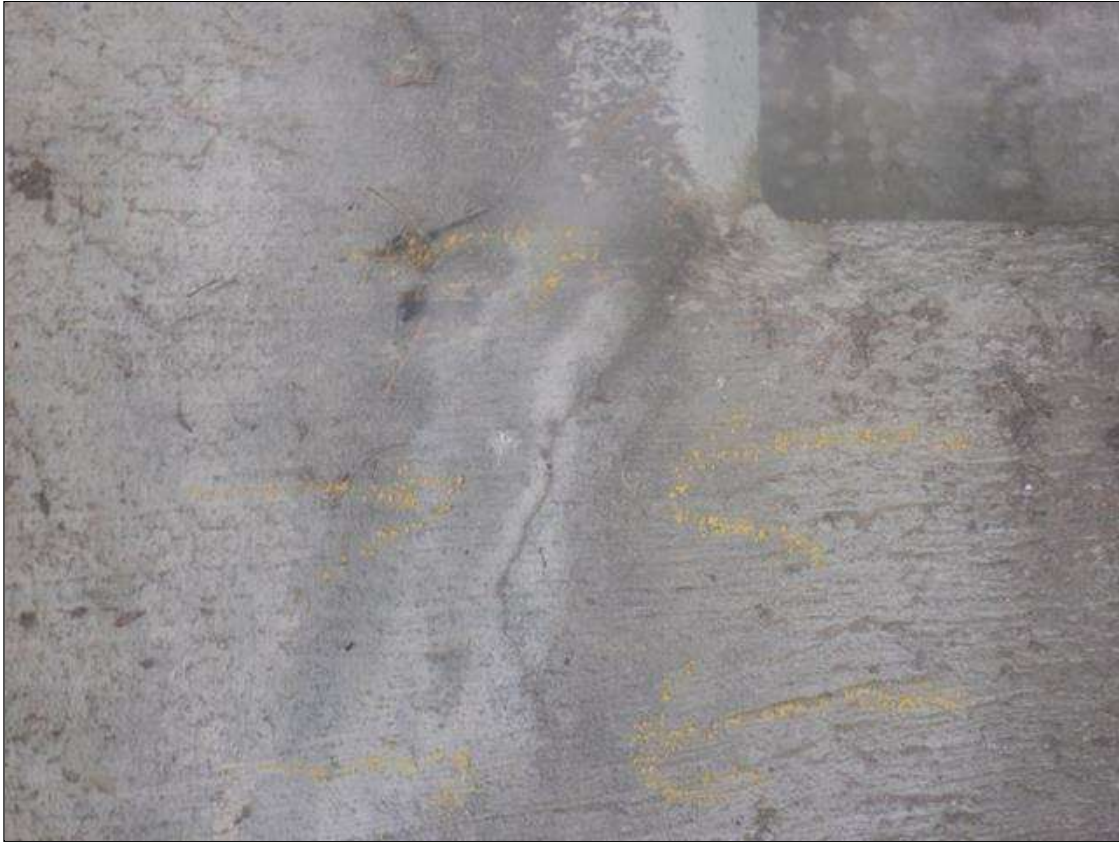
End Bent 2 Cap 1: (2) UP TO 12" X 1/64" DIAGONAL CRACKS, SOUTH FACE, EXTENDING FROM EAST AND WEST SIDES OF BEAM 4 BEAM SEAT.
