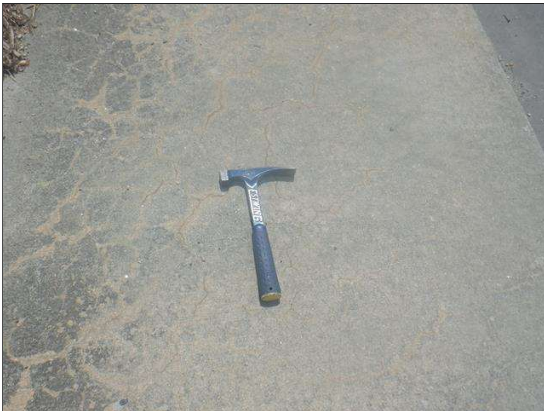
Span 3 Deck: MAP CRACKING WITH EFFLORESCENCE UP TO 1/64 IN WIDE SCATTERED ALONG THE LENGTH OF THE SIDEWALK
