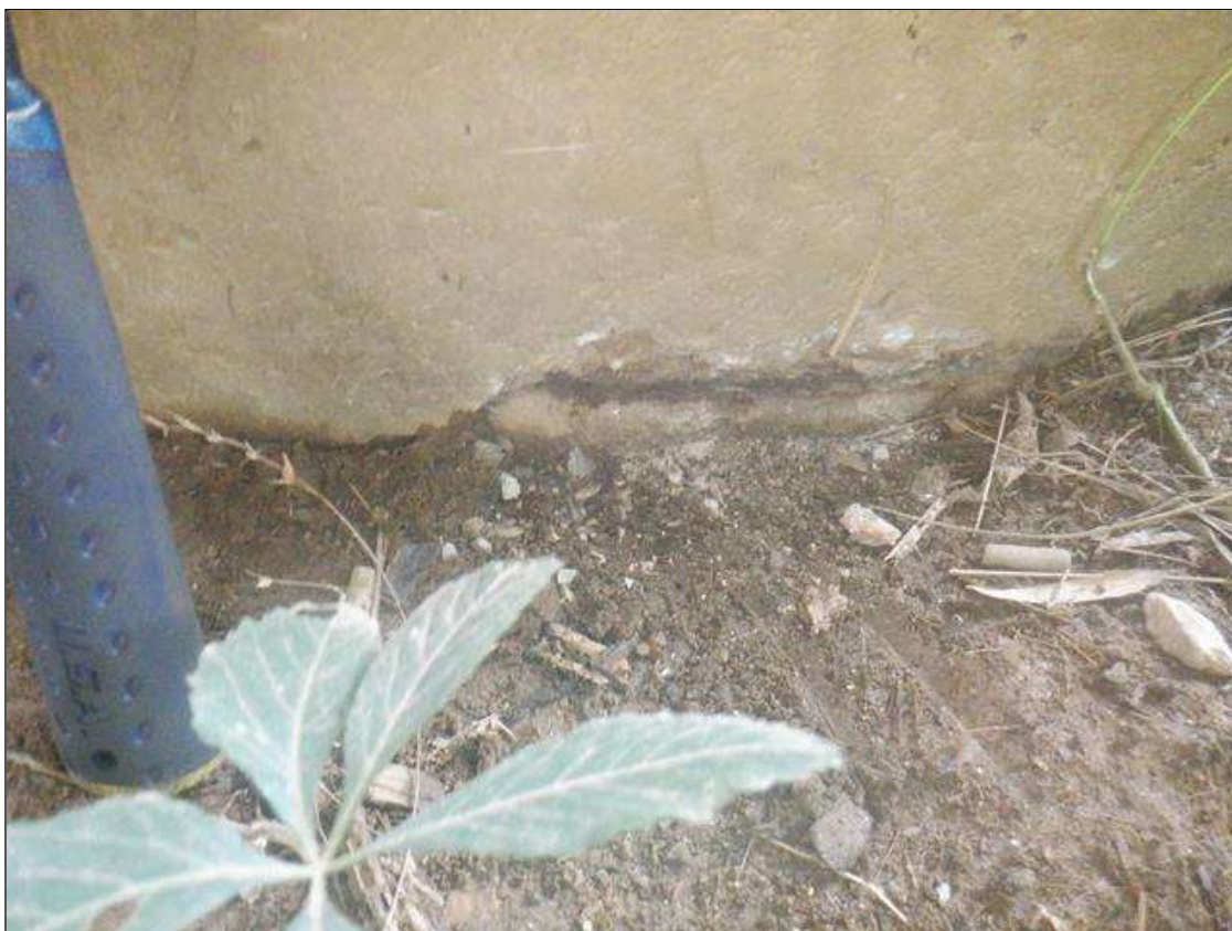
Bent 3 Pile 3: 10 IN LONG X UP TO 3 IN WIDE X 1/2 IN DEEP SPALL, WITH EXPOSED REINFORCING, WEST FACE AT GROUND LEVEL
