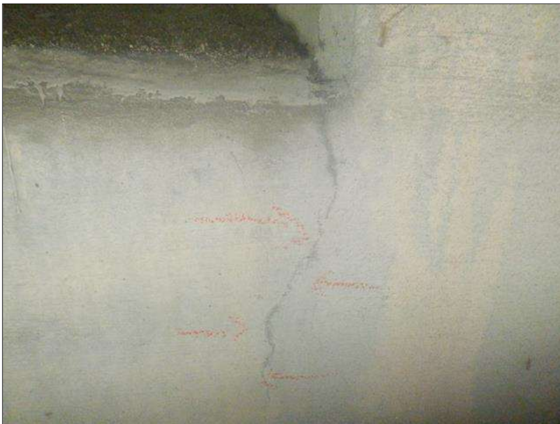
End Bent 1 Cap 1: 12 IN LONG X 1/64 IN WIDE VERTICAL CRACK, NORTH FACE, BETWEEN BEAMS 3 AND 4, NEAR BEAM 3.
