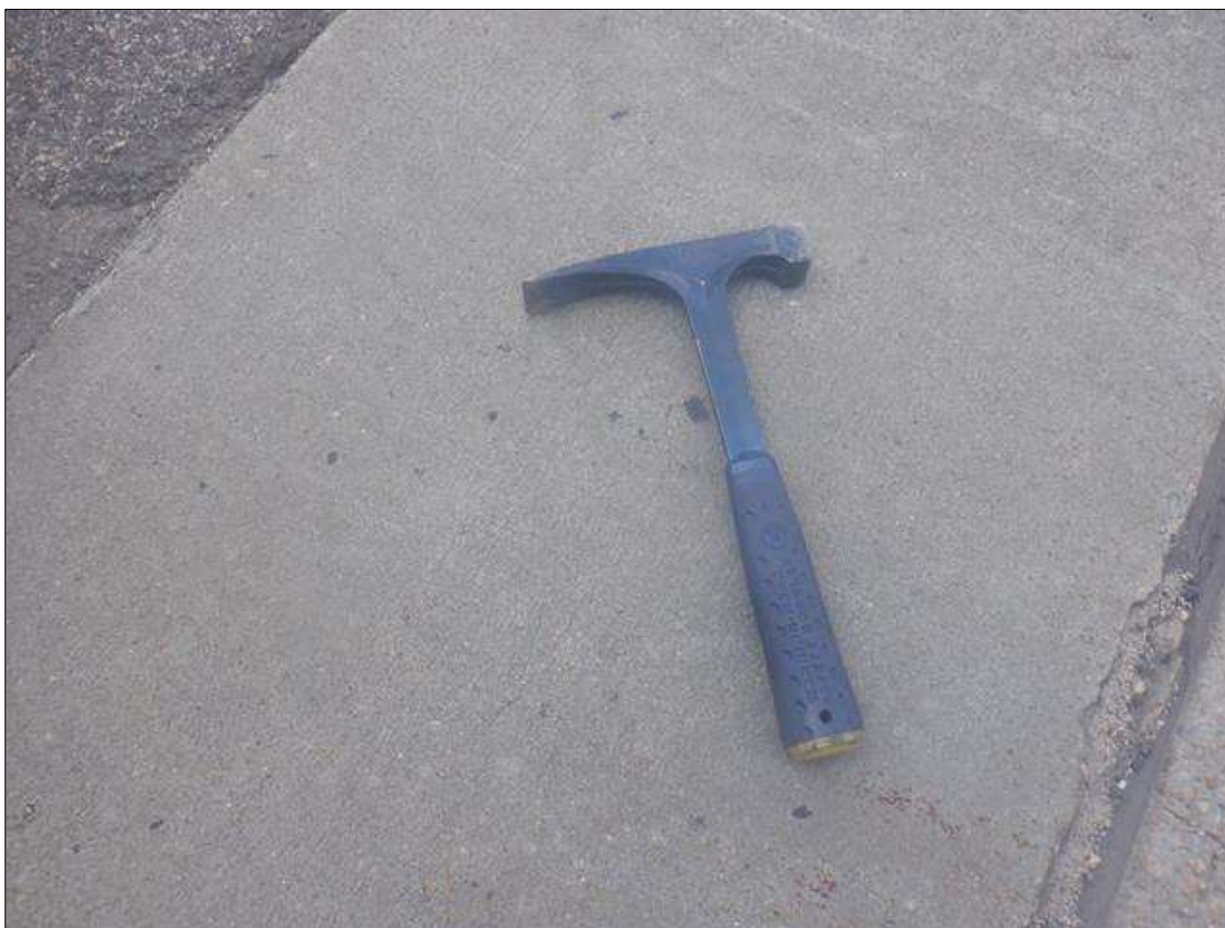
Approach 1 : HAIRLINE MAP CRACKING ALONG FULL LENGTH OF APPROACH.
