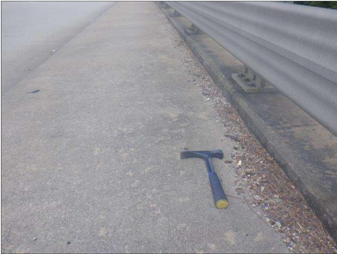
MINOR DECK DEBRIS ALONG THE EDGE OF THE SIDEWALK IN ALL SPANS
