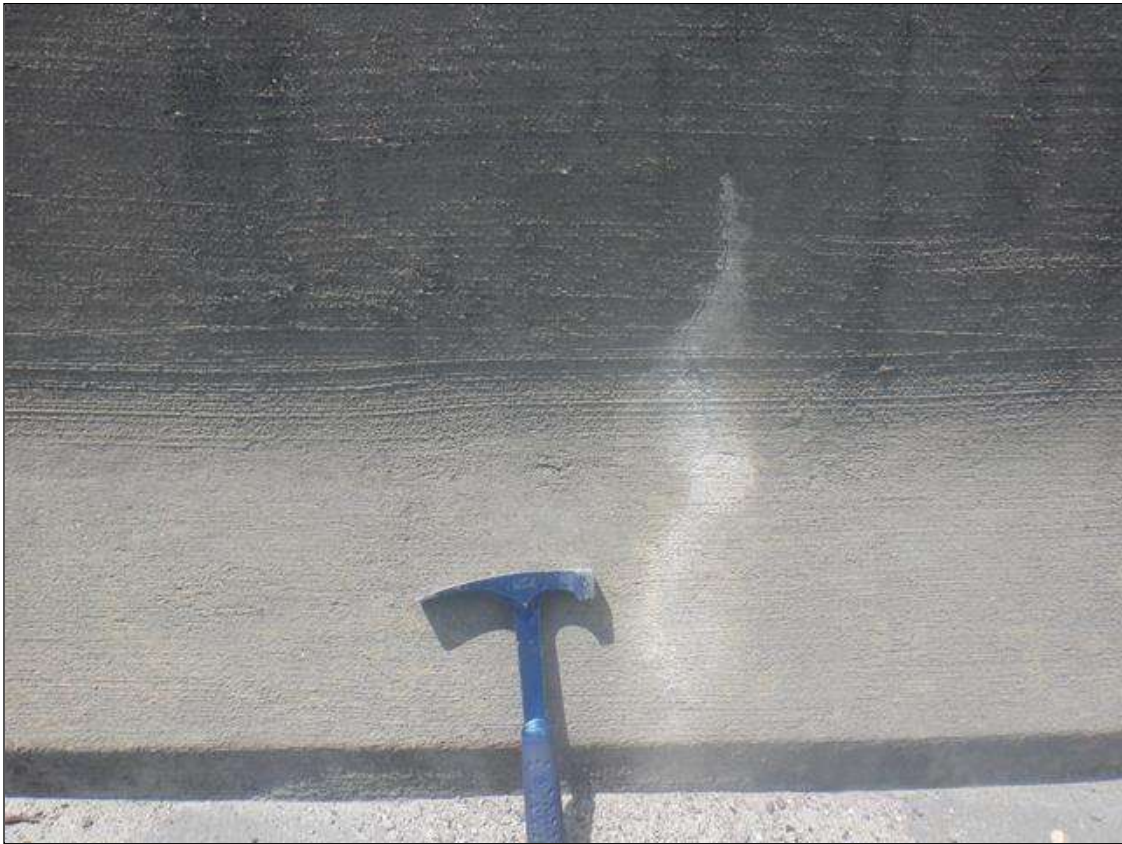
Span 1 Left Bridge Rail: (7) UP TO 1/32 IN WIDE WRAP-AROUND CRACKS, WITH EFFLORESCENCE, AT RANDOM THROUGHOUT.
