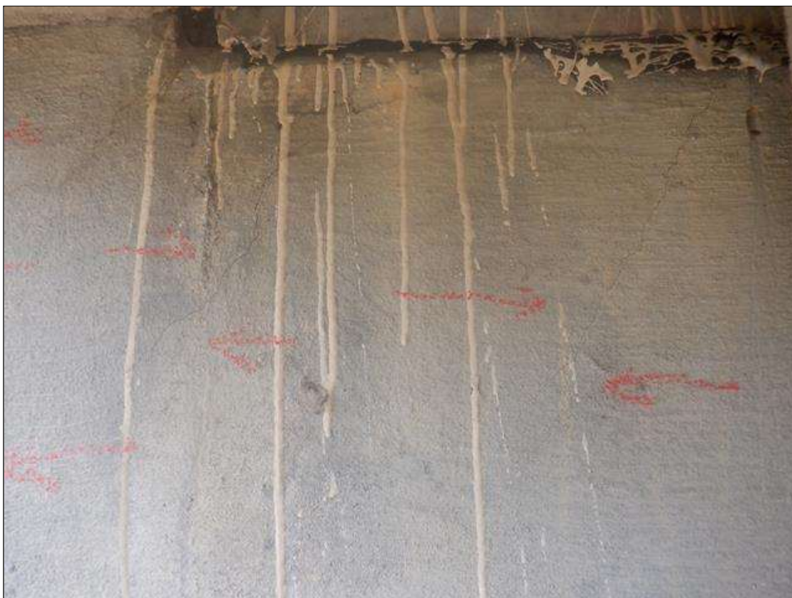
End Bent 2 Abutment: THREEE (3) UP TO 2 FT LONG X 1/64 IN WIDE DIAGONAL CRACKS TO THE LEFT OF BEAM 1 NEAR THE TOP OF THE WALL
