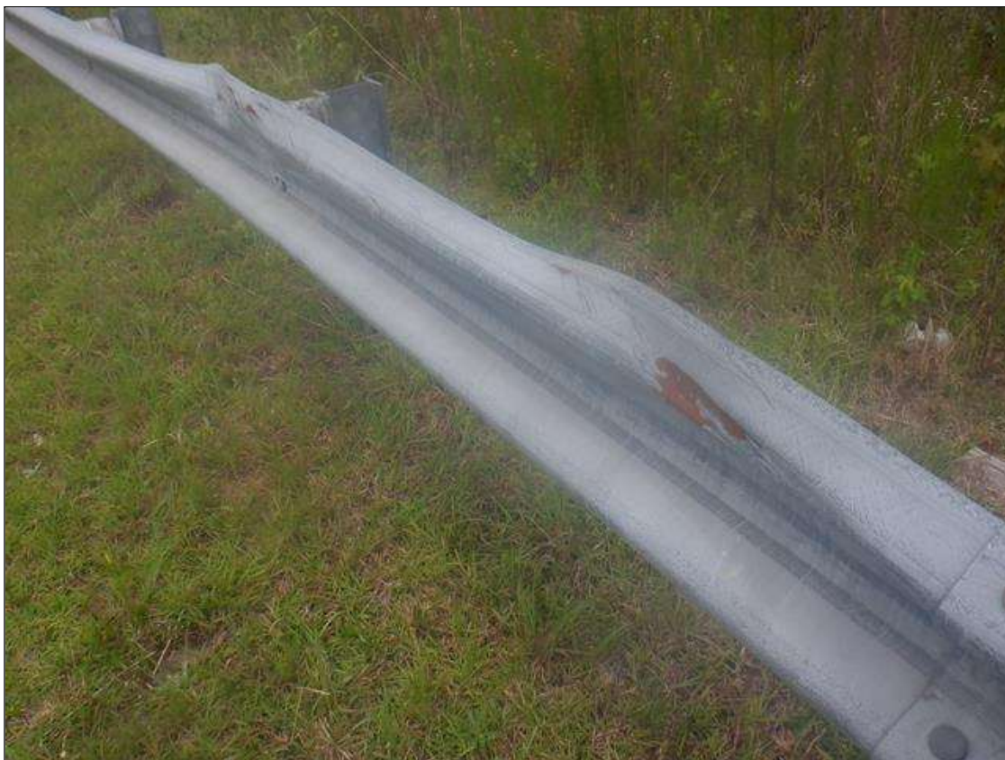
MODERATE IMPACT DAMAGE TO NORTHEAST GUARDRAIL AT MID SPAN FOR UP TO 13 FT LONG WITH RAIL DEFLECTED INWARD FOR 4 INCHES. (PAR)
