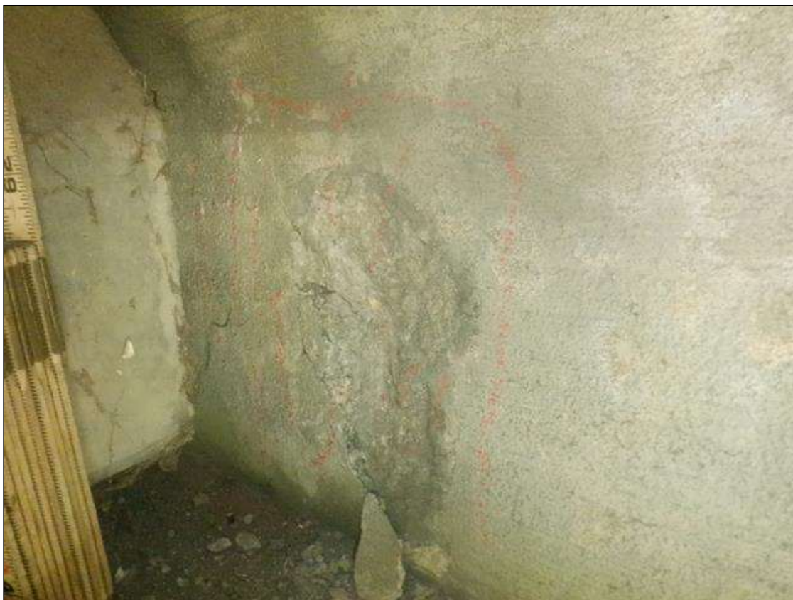
End Bent 2 Cap 1: UP TO 10 IN WIDE X 8 IN HIGH X UP TO 3/4 IN DEEP SPALL TO THE RIGHT SIDE OF BEAM 2 BOTTOM FLANGE
