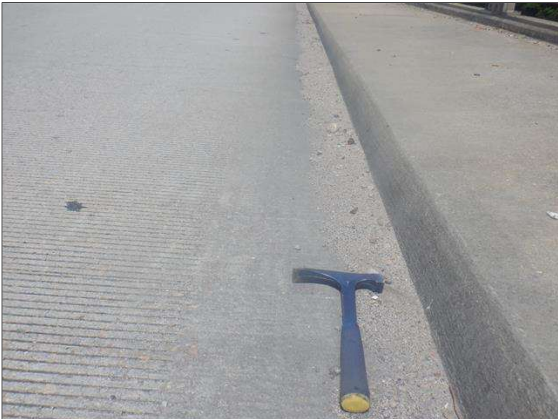
MINOR DECK DEBRIS ALONG THE RIGHT CRUB AND LEFT BRIDGE RAIL IN ALL SPANS
