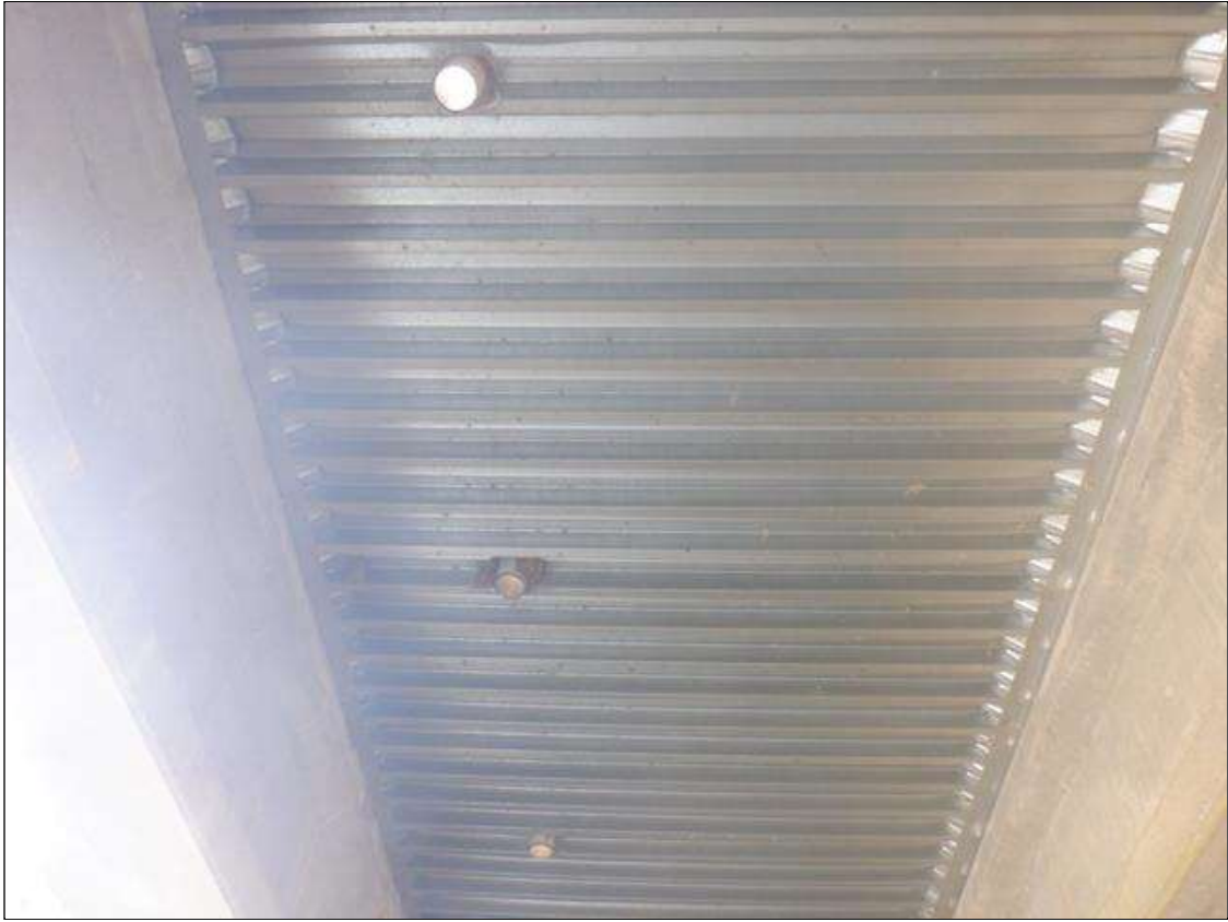
TYPICAL DRAINAGE PIPES IN SPAN 3 BAY 4
