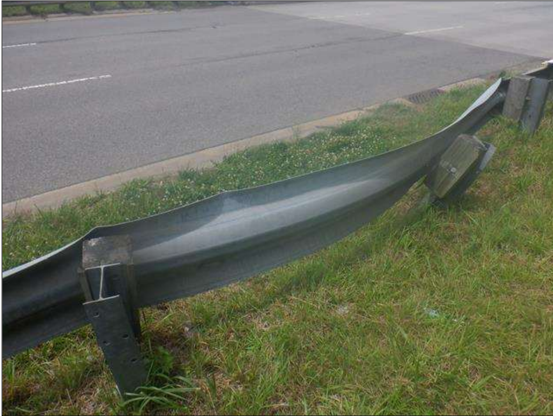
HEAVY IMPACT DAMAGE TO SOUTHEAST GUARDRAIL FOR 13 FROM LONG STARTING 24 FT FROM BEGINNING OF BRIDGE. RAIL IS DEFLECTED INWARD UP TO 24 INCHES AND VERTICAL POST ARE LEANING EAST AND TWISTED. (PAR)
