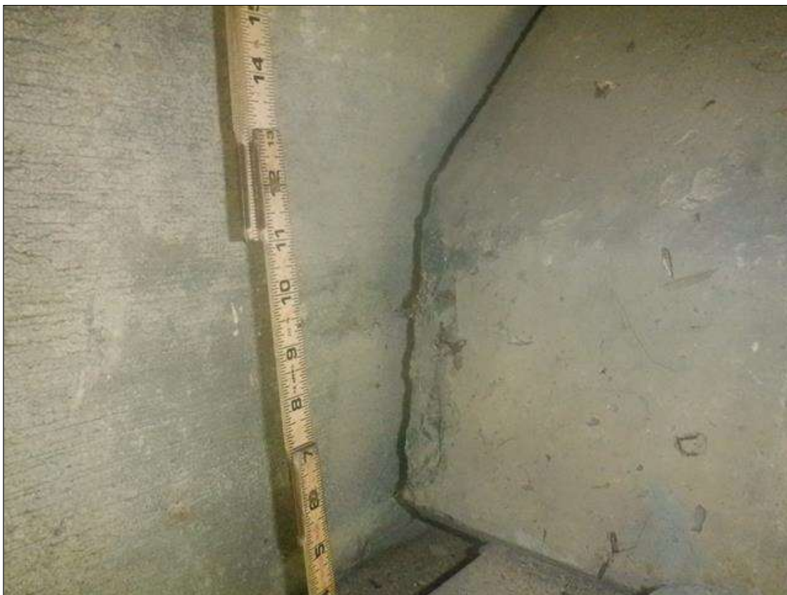
Span 1 Beam 2: RIGHT BOTTOM FLANGE AT ABUTMENT 1, SPALL APPROXIMATELY 2 IN LONG X 8 IN HIGH X UP TO 3/4 DEEP
