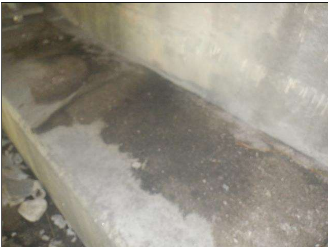
DEBRIS ON TOP OF THE CAP FOR FULL LENGTH
