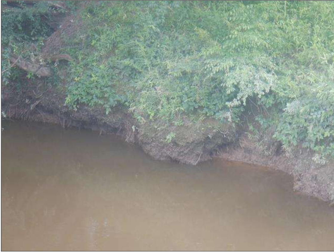
SLUMPING UP TO 40 FT LONG X 2 FT HIGH X 1 FT DEEP IN THE RIGHT BANK AT THE DOWNSTREAM END, STARTING 50 FT FROM THE BRIDGE
