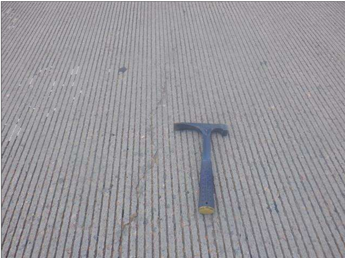
Span 1 Deck: SCATTERED TRANSVERSE CRACKING TO 1/16" WIDE AT AVERAGE 6' SPACING FOR FULL WIDTH.
