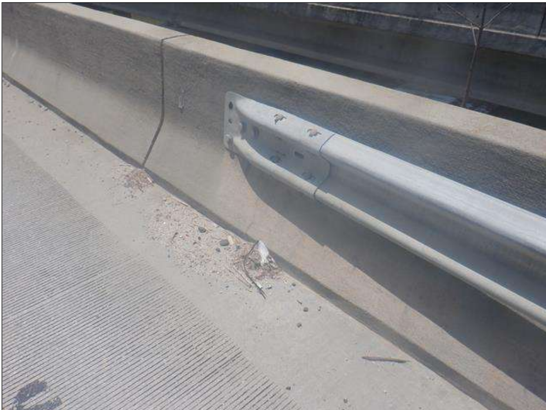
GUARDRAIL TO BRIDGE RAIL CONNECTION AT NORTHWEST CORNER. SIMILAR AT SOUTHWEST CORNER
