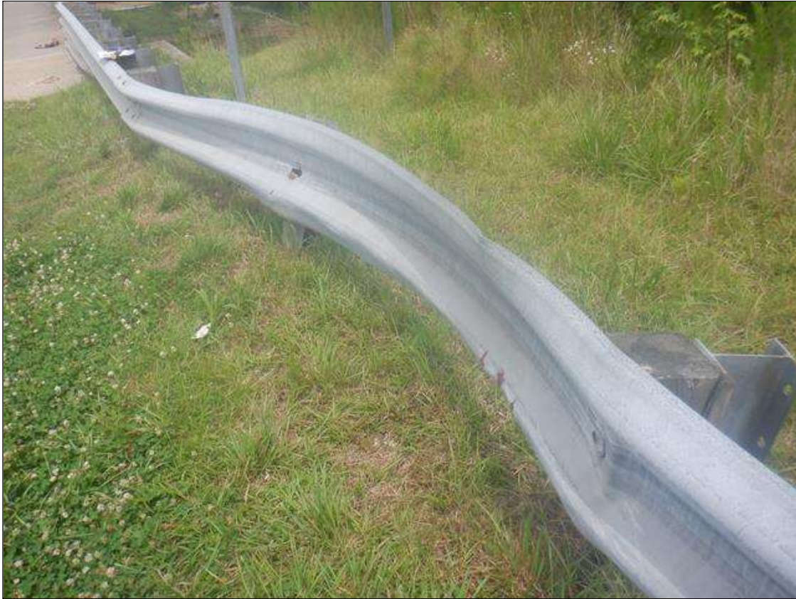
HEAVY IMPACT DAMAGE TO SOUTHEAST GUARDRAIL FOR 13 FROM LONG STARTING 24 FT FROM BEGINNING OF BRIDGE. RAIL IS DEFLECTED INWARD UP TO 24 INCHES AND VERTICAL POST ARE LEANING EAST AND TWISTED. (PAR)
