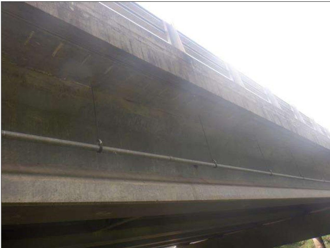
3 IN DIAMETER UTILITY PIPE IN RIGHT OVERHANG.
