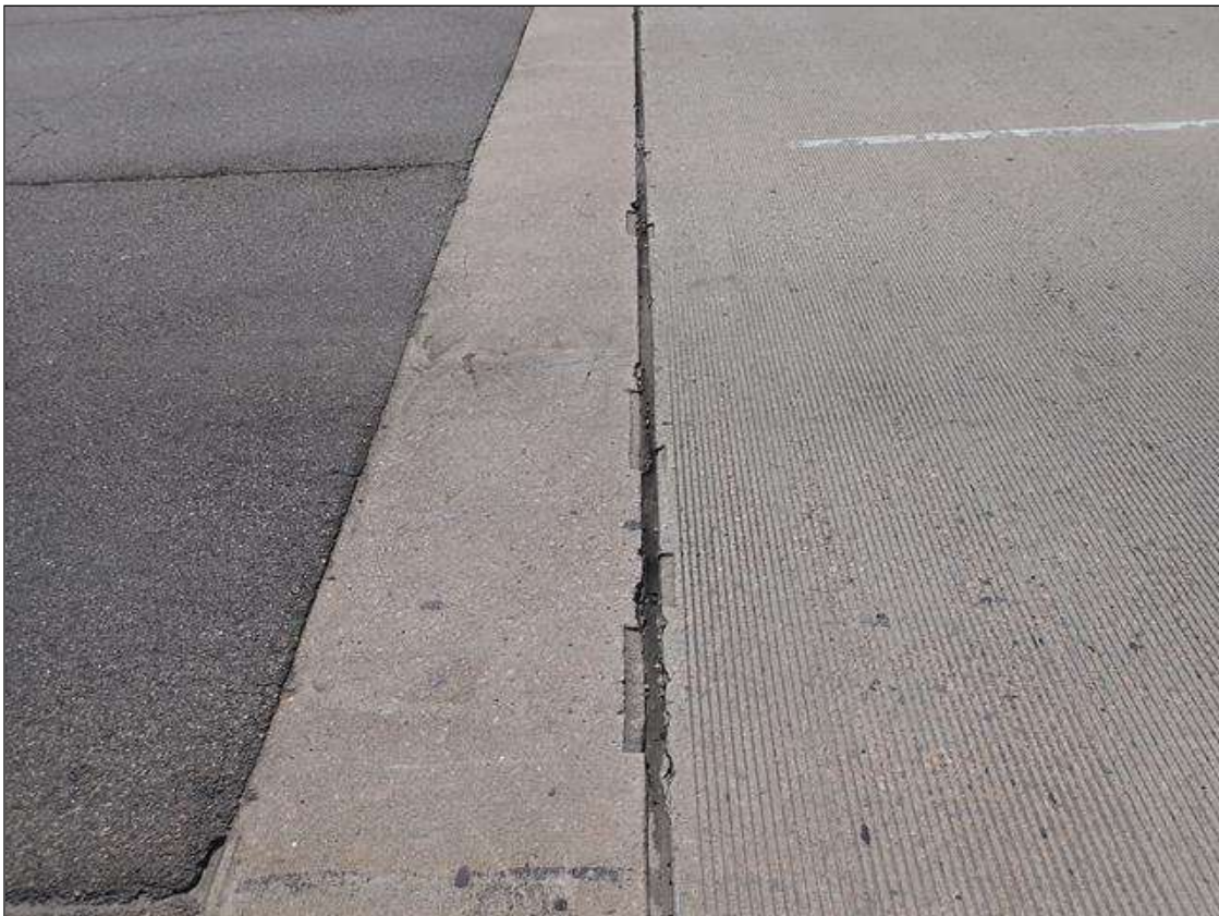
Span 4 Expansion Joint 5: NUMEROUS SOUND PATCHES UP TO 1 FOOT LONG X 2 INCHES WIDE AT VARIOUS LOCATIONS BOTH SIDES OF JOINT
