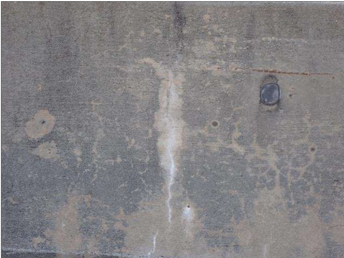
Span 1 Right Bridge Rail: BOTH FACES SCATTERED THROUGHOUT, VERTICAL CRACKS (FULL HEIGHT X HAIRLINE) WITH EFFLORESCENCE EXTENDING ONTO TOP FACE (FULL WIDTH X UP TO 1/32 INCH)
