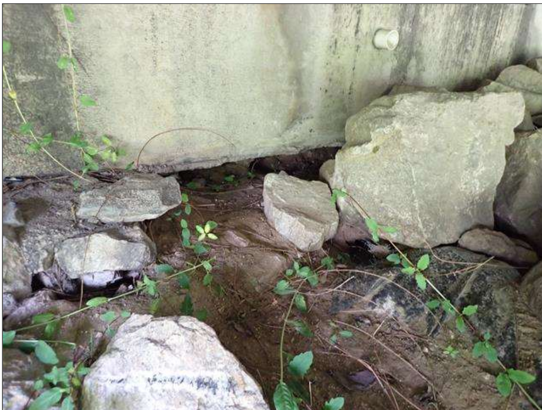
End Bent 2 Abutment: BAY 2, AREA OF MISSING RIP RAP WITH VOID (5 FEET X UP TO 9 INCHES) NO UNDERMINING
