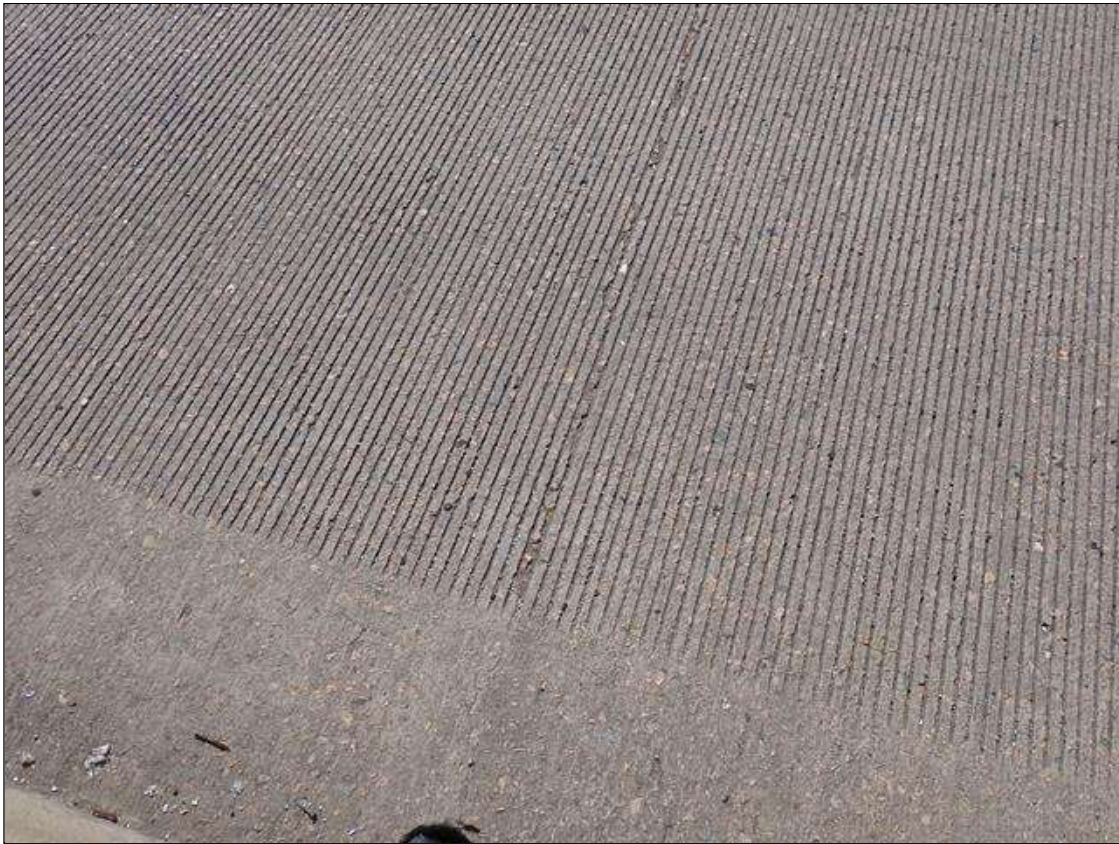
Span 1 Deck: SEVERAL FULL/PARTIAL WIDTH TRANSVERSE CRACKS UP TO 1/32 INCH AT VARIOUS LOCATIONS IN TOP OF DECK
