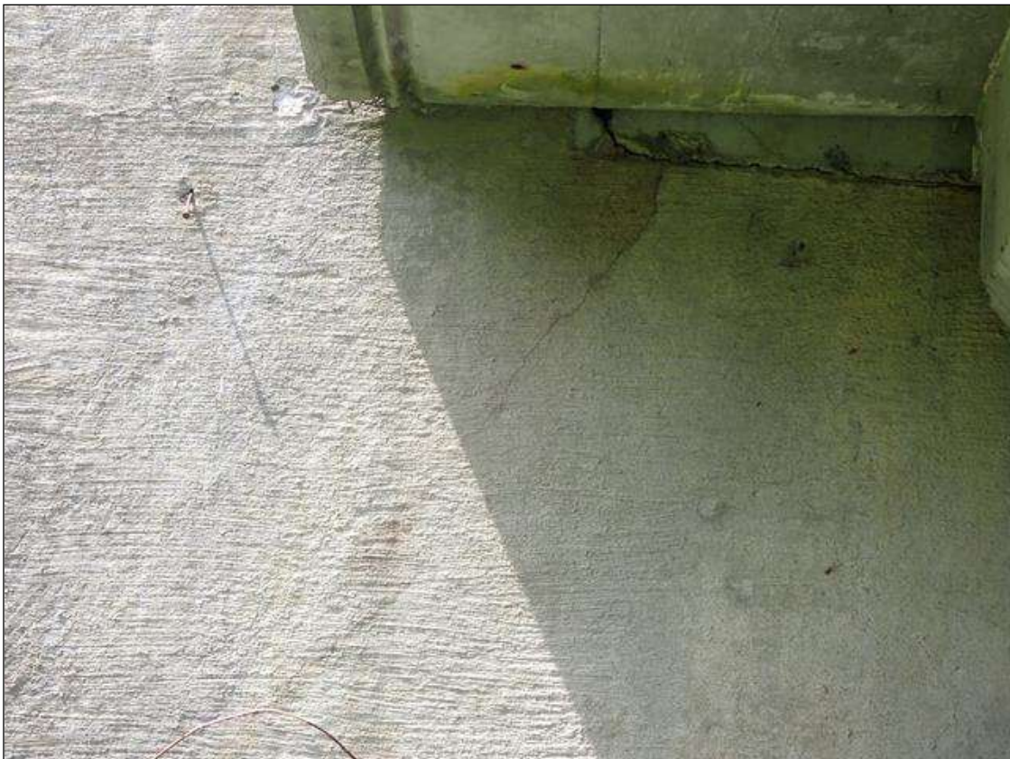
End Bent 1 Abutment: EAST END OF ABUTMENT, 4 FOOT LONG DIAGONAL 1/32 INCH CRACK
