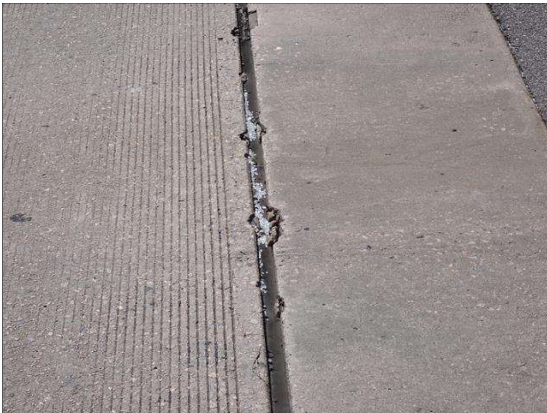
Span 1 Expansion Joint 1: ALL LANES SCATTERED THROUGHOUT, EDGE SPALLING (UP TO 18 INCHES X 2 INCHES X 1/2 INCH) NO EXPOSED REBAR
