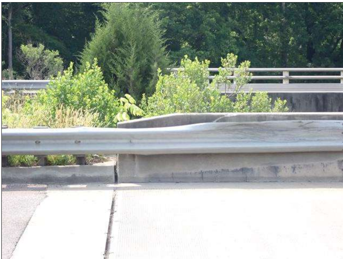
AT NORTHEAST CORNER OF BRIDGE, IMPACT DAMAGE TO APPROACH GUARDRAIL FOR 6 FEET WITH RAIL DEFLECTED DOWN UP TO 2 INCHES, GUARDRAIL IS FUNCTIONING AS INTENDED
