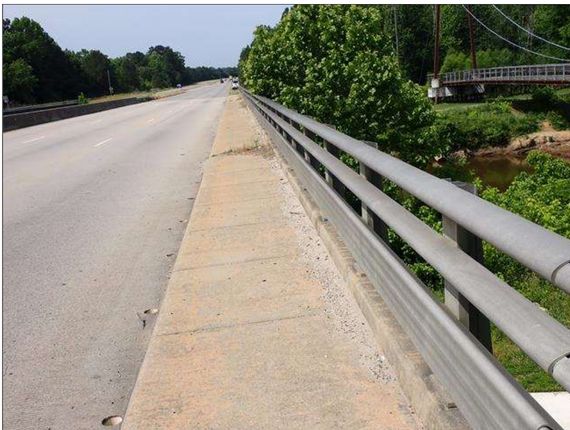
DEBRIS OVER BENT 3 JOINT
