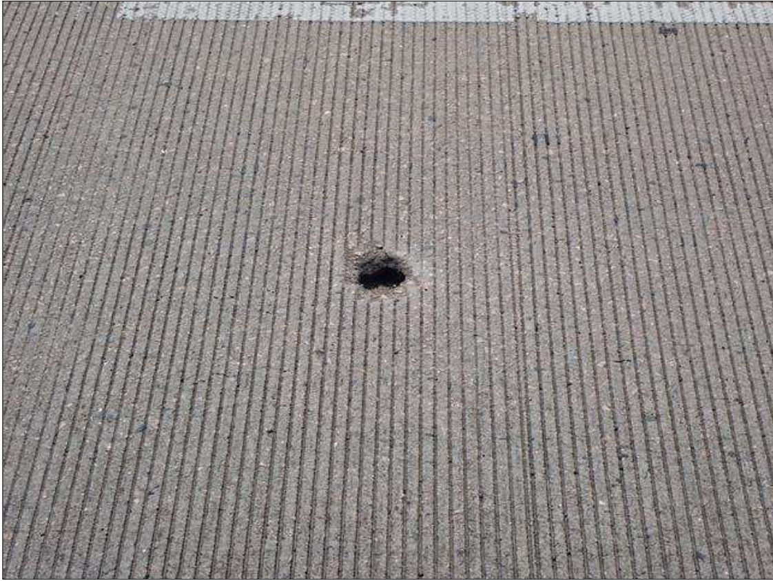
Span 3 Deck: IN LEFT TRAVEL LANE, BORE HOLE (3 INCH DIAMETER X UP TO 1-1/2 INCH DEEP) NO EXPOSED REBAR
