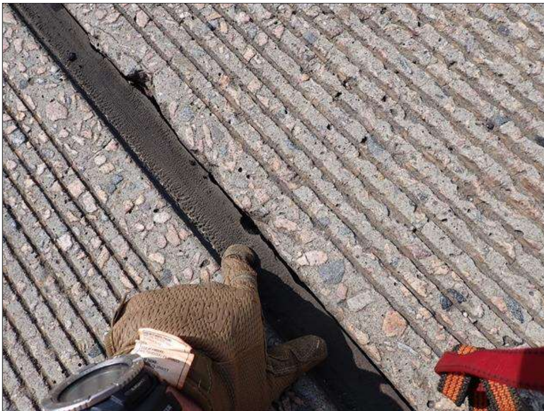
Span 3 Expansion Joint 3: IN LEFTMOST LANE, PARTIAL DEPTH ADHESION LOSS
