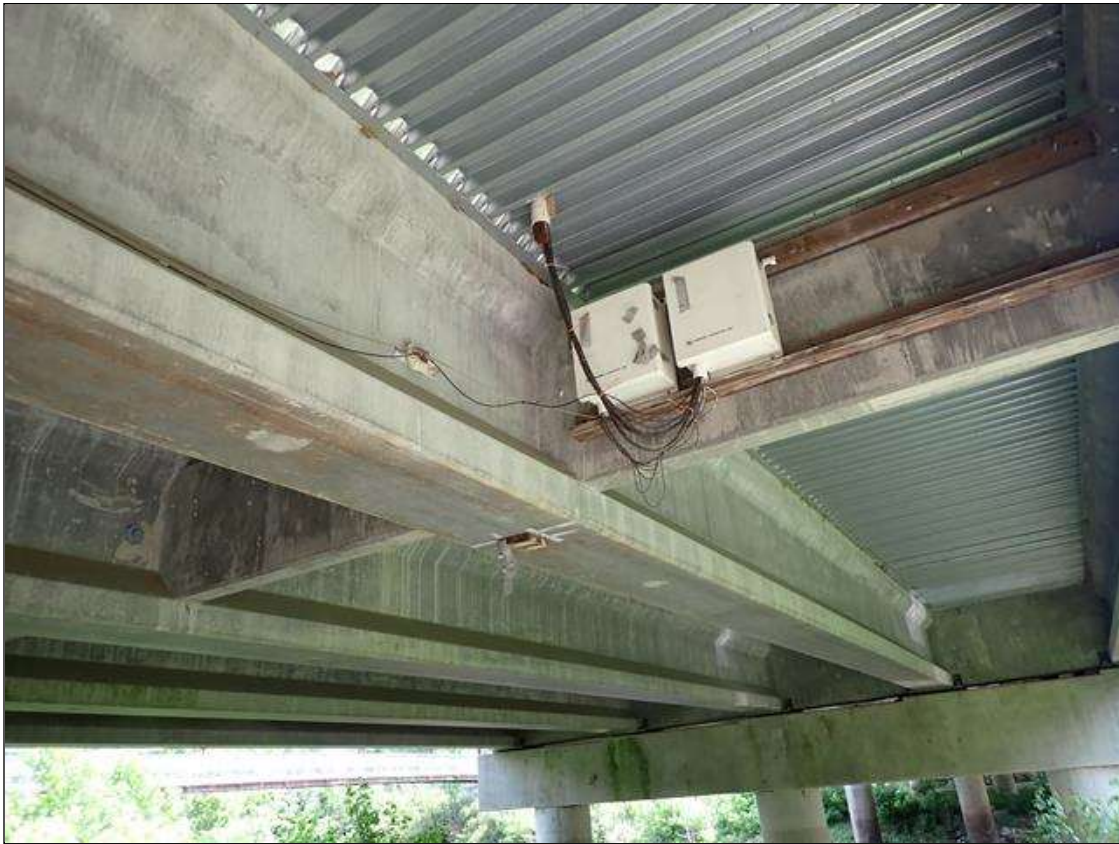
MONITORING EQUIPMENT ATTACHED TO SPAN 1 BAY 4 INTERMEDIATE DIAPHRAGM
