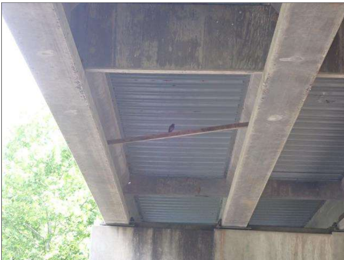
BOARDS WEDGED BETWEEN GIRDERS IN BAYS 1 AND 4 OF SPAN 2, 3 TOTAL
