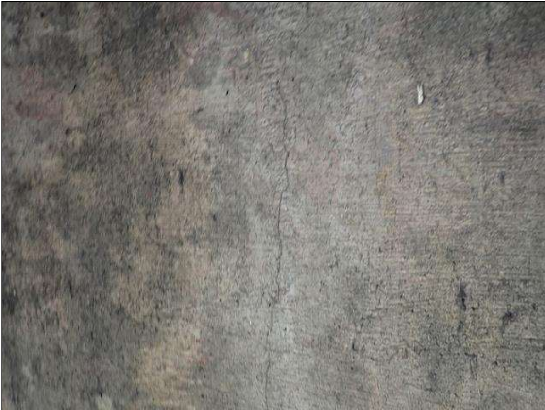
End Bent 1 Abutment: VERTICAL HAIRLINE CRACKS IN THE BACKWALL BETWEEN GIRDERS
