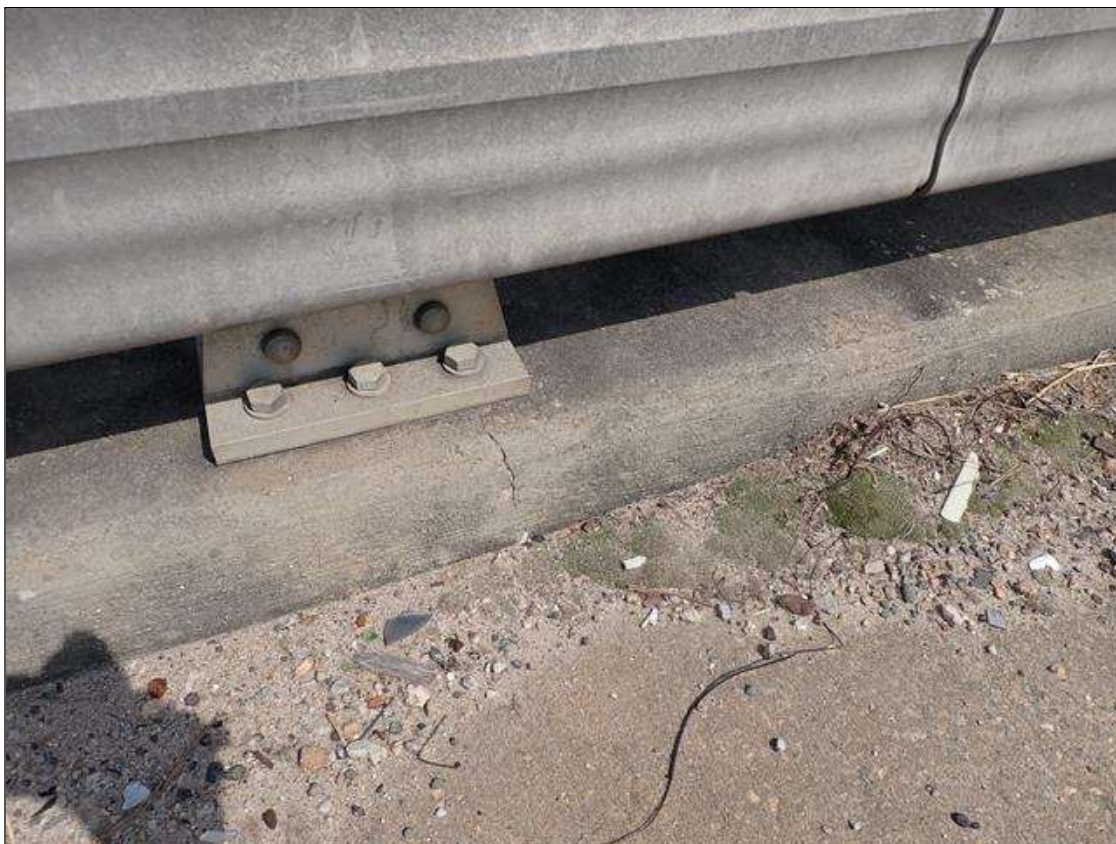
Span 2 Left Bridge Rail: BOTH FACES AND TOP OF PARAPET AT APPROXIMATELY 5 FOOT CENTERS, VERTICAL HAIRLINE CRACKS UP TO 1 FOOT HIGH, SOME WITH EFFLORESCENCE
