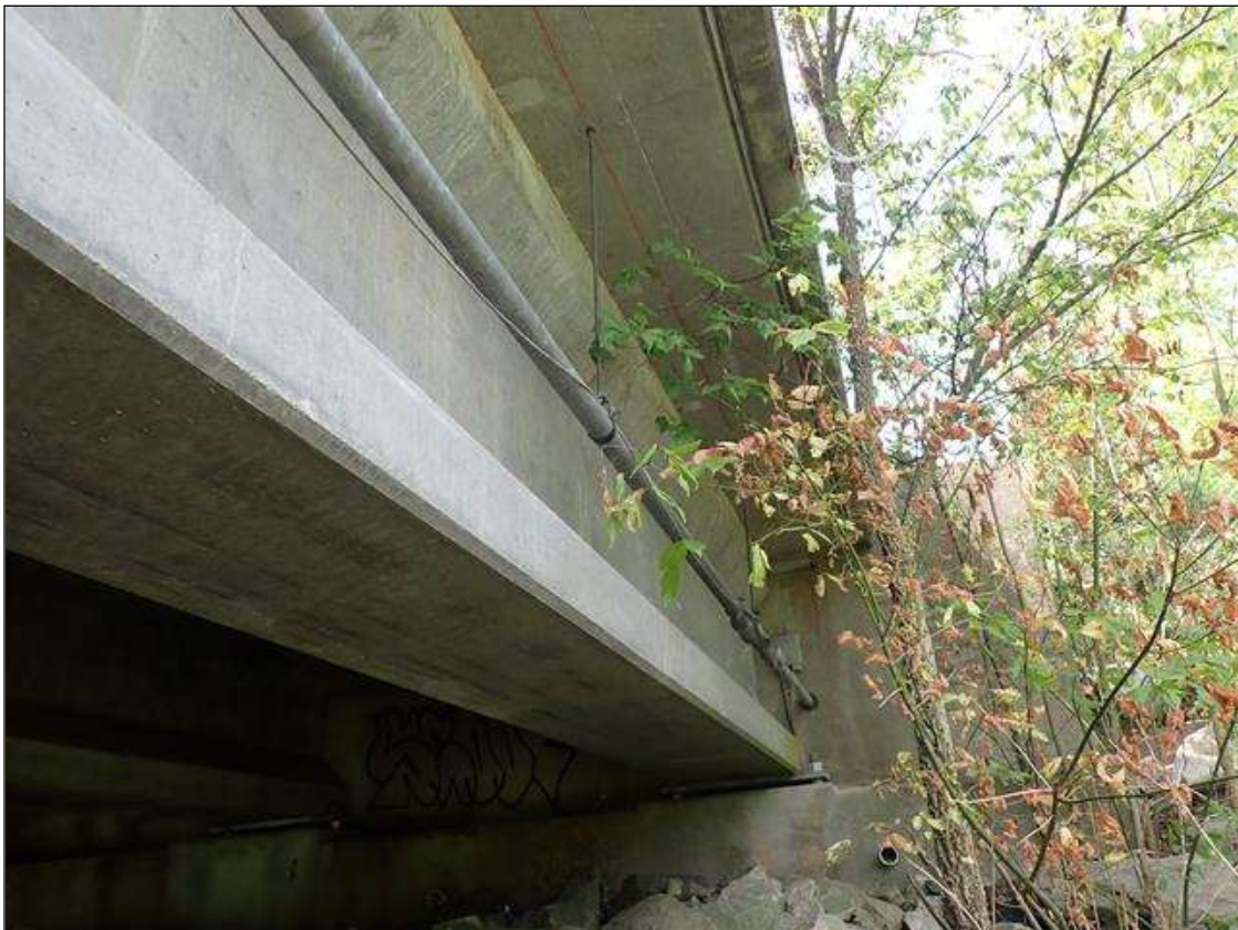
UTILITY IN WEST OVERHANG
