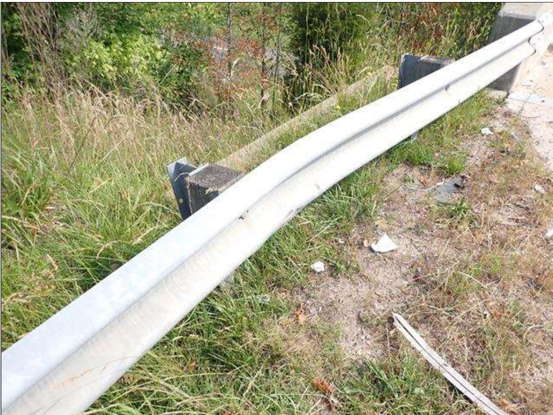
STARTING AT SOUTHWEST CORNER OF BRIDGE, IMPACT DAMAGE TO APPROACH GUARDRAIL FOR 10 FEET WITH POSTS ROTATED AND PUSHED BACK UP TO 1 FOOT, GUARDRAIL IS FUNCTIONING AS INTENDED
