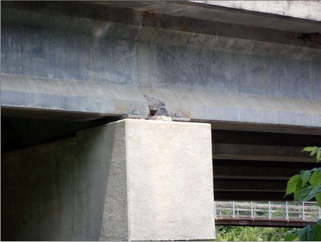
END DIAPHRAGM AT BENT 1 BEAM END, SPALL (1 FOOT TALL X 9 INCHES LONG X UP TO 4 INCHES DEEP) WITH EXPOSED RUSTED REBAR, NO MEASURABLE SECTION LOSS
