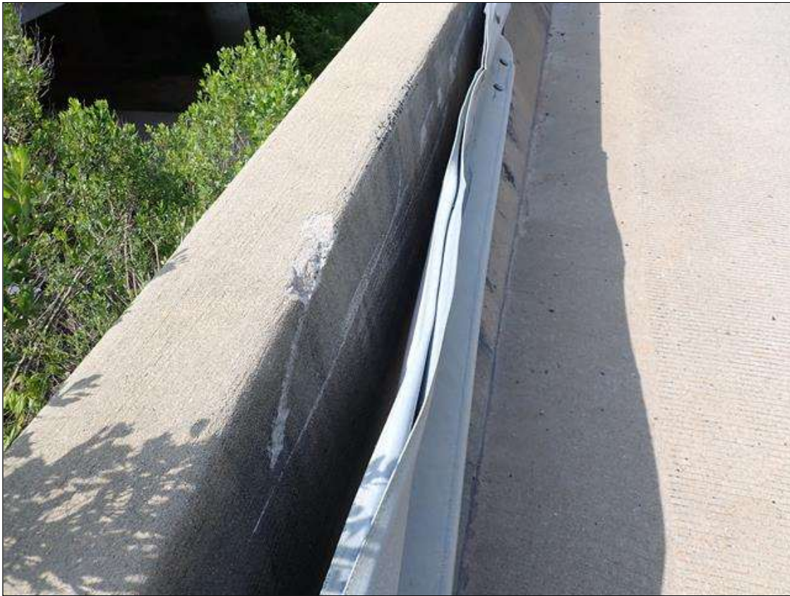
Span 4 Right Bridge Rail: TOP OF RAIL AT END BENT 2, SPALL (6 INCHES LONG X 1 INCH TALL X 1/2 INCH DEEP) NO EXPOSED REBAR
