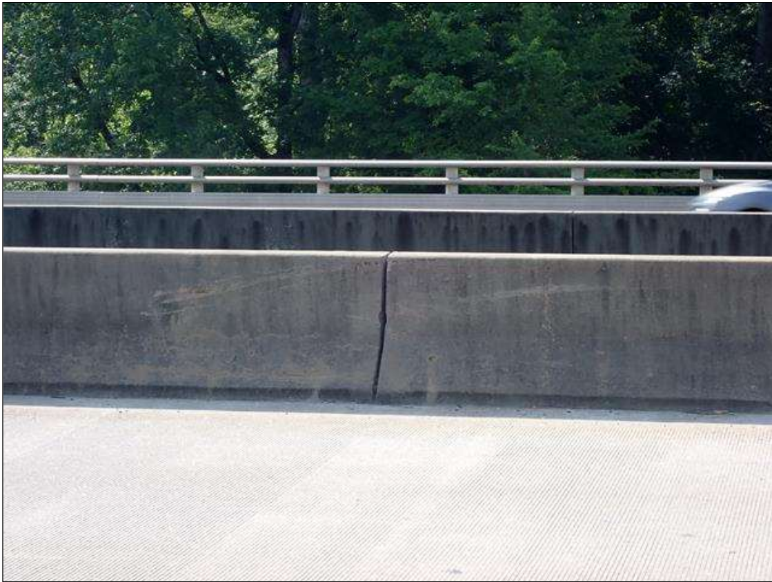
TYPICAL IMPACT SCRAPE IN RIGHT BRIDGE RAIL, NO SECTION LOSS
