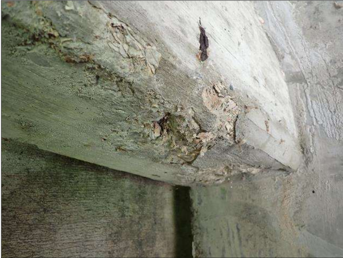
Span 1 Beam 4: IN END BENT END DIAPHRAGM NEAR RIGHT TOP FLANGE, EXPOSED REBAR AND ROTTEN CONCRETE WITH NO STRENGTH FALLING APART (14 INCHES WIDE X 7 INCHES HIGH X 2 INCHES LONG X UP TO 1/2 INCH DEEP) NO REBAR EXPOSED BELOW FAULTY CONCRETE
