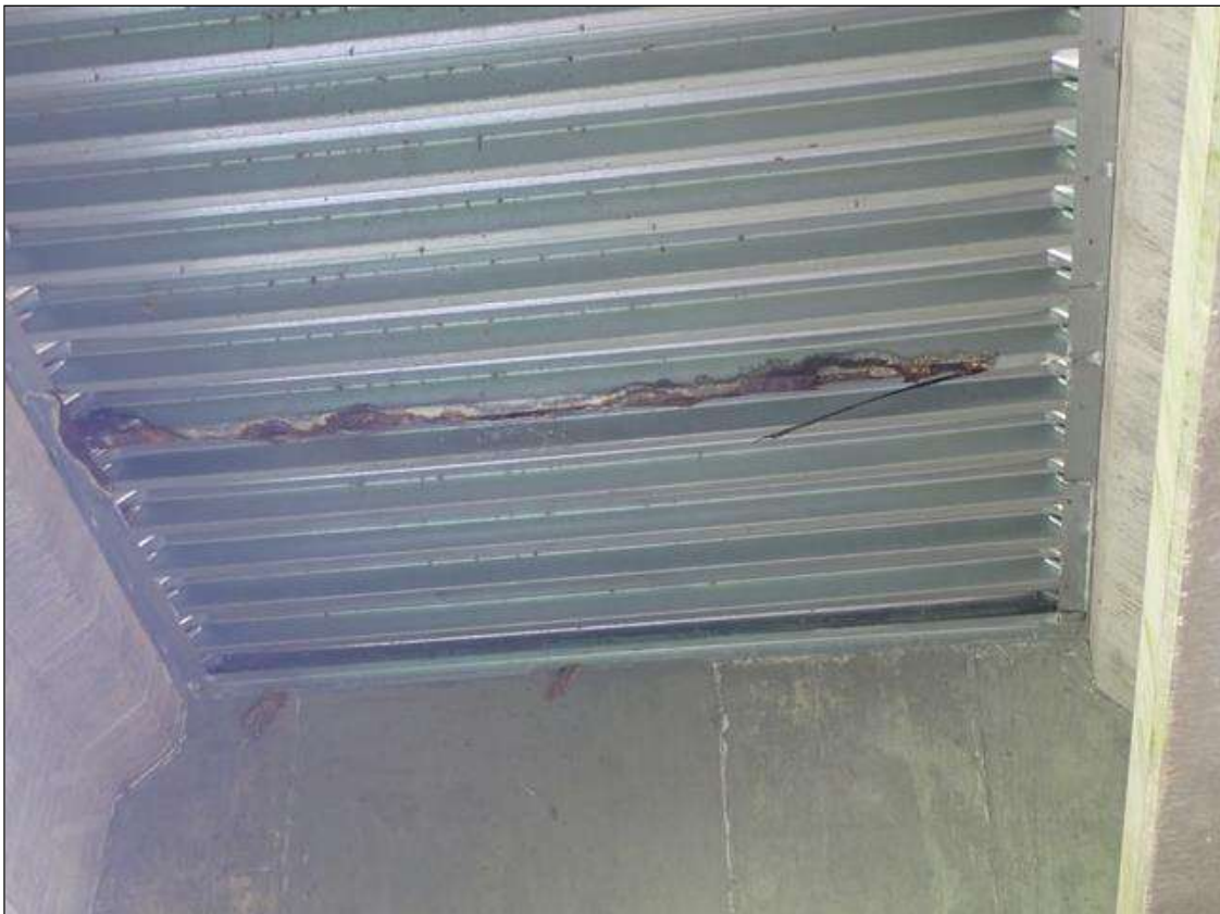
Span 1 Deck: 4 FEET FROM BENT 1 IN BAY 1, CORROSION ON STAY IN PLACE FORM (8 FEET WIDE X 8 INCHES LONG)
