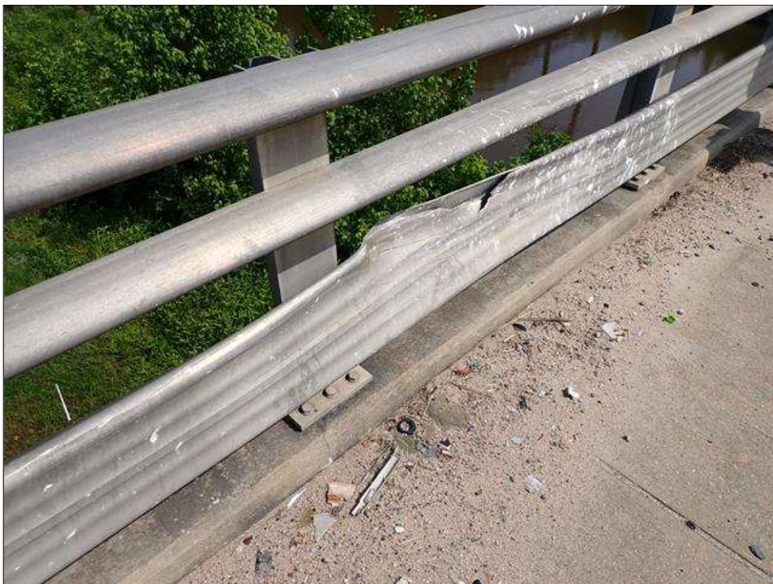
Span 1 Left Bridge Rail: AT 45 FEET FROM END BENT 1, IMPACT DAMAGE BOTTOM RAIL (3-1/2 LINEAR FEET) WITH TEARING (30 INCHES X UP TO 3 INCHES) NO DAMAGE TO POSTS
