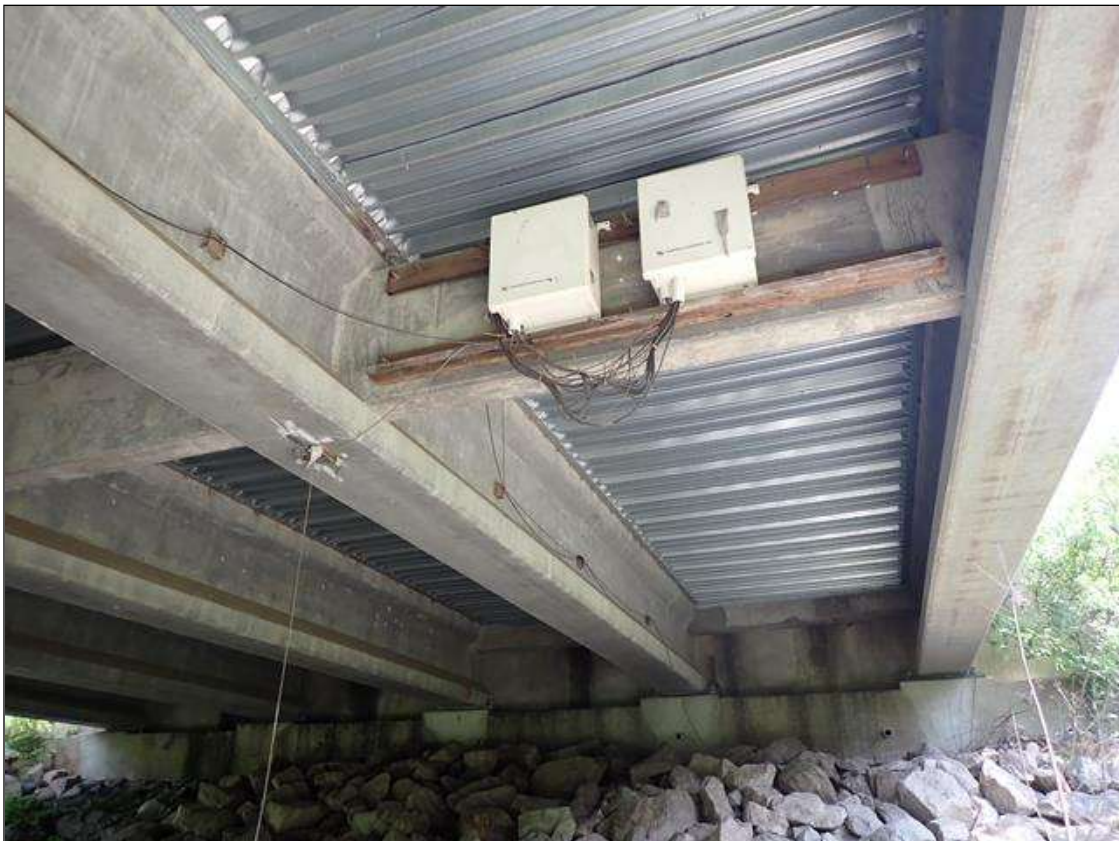
MONITORING EQUIPMENT ATTACHED TO SPAN 4 BAY 3 INTERMEDIATE DIAPHRAGM
