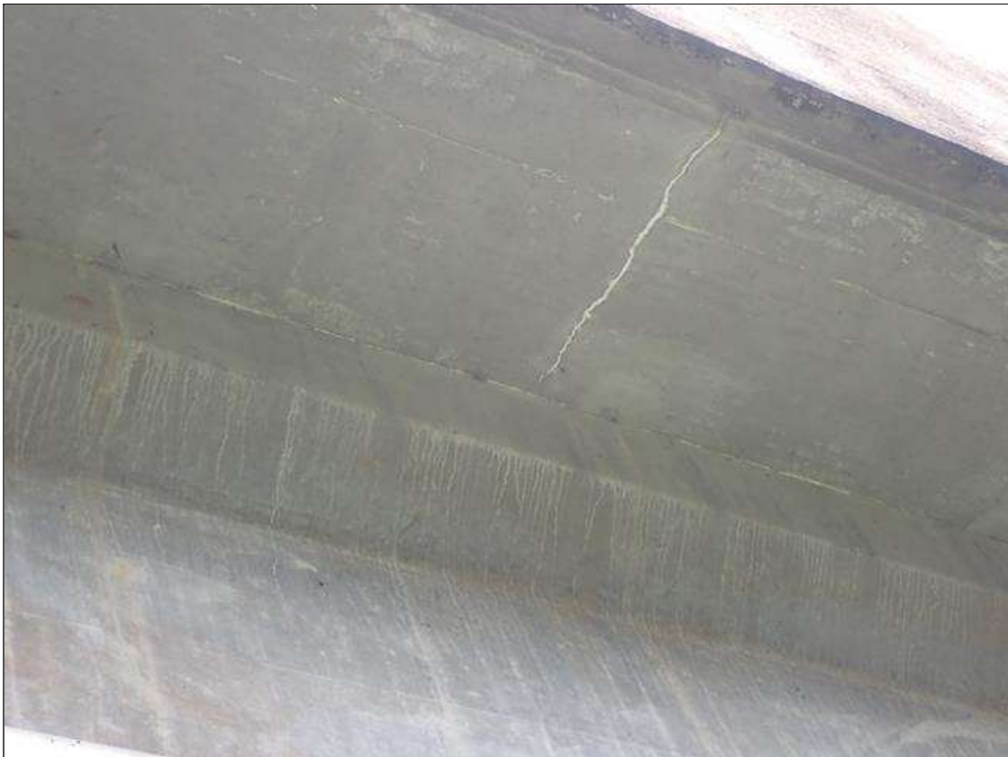
Span 1 Deck: EAST OVERHANG SCATTERED THROUGHOUT, TRANSVERSE CRACKS (2 FEET X HAIRLINE) WITH EFFLORESCENCE
