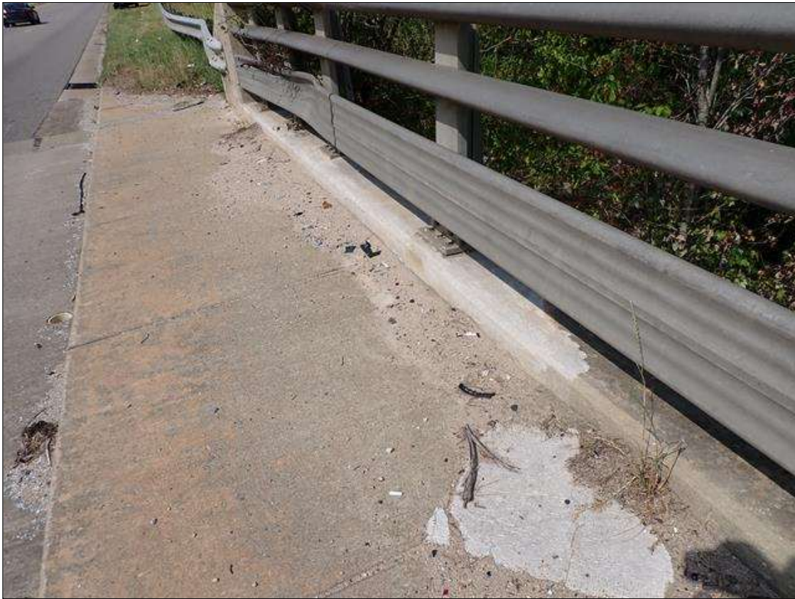
Span 1 Left Bridge Rail: PARAPET AT END BENT 1, REPAIR AREA (13 LINEAR FEET)
