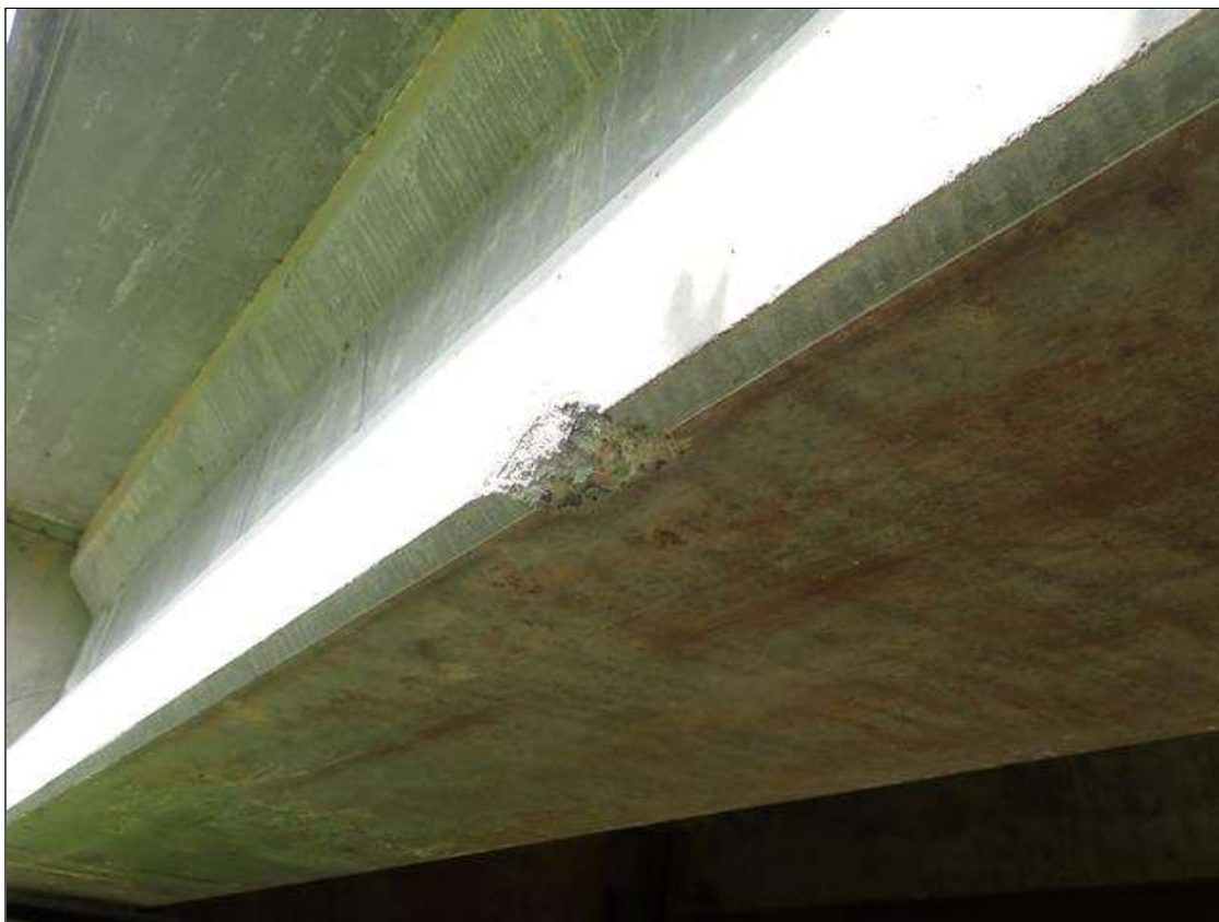
Span 1 Beam 5: 8 FEET FROM ABUTMENT 1 IN BOTTOM FLANGE ON BOTTOM EAST CORNER, SPALL (4 INCHES X 3 INCHES X 1 INCH DEEP) NO EXPOSED REBAR
