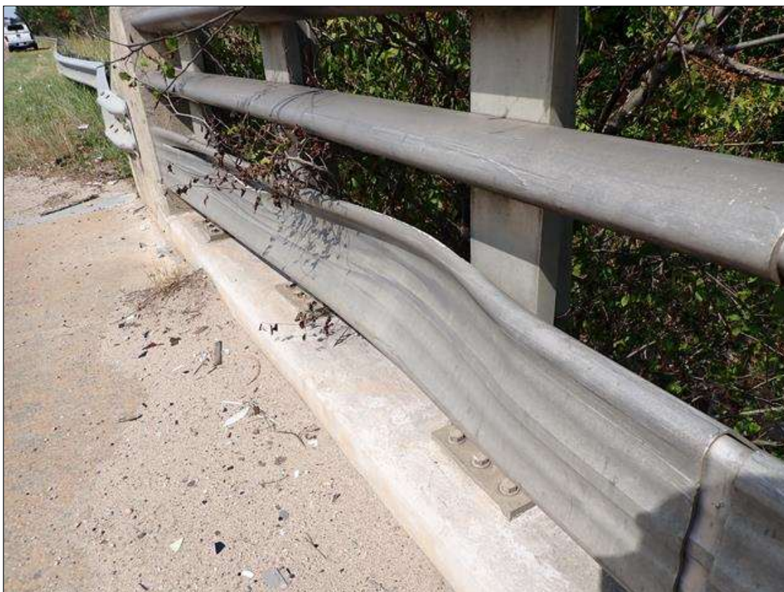
Span 1 Left Bridge Rail: AT END BENT 1, IMPACT DAMAGE TO BOTTOM RAIL (9-1/2 LINEAR FEET) WITH TEARING (5 FEET X UP TO 2 INCHES) NO DAMAGE TO POSTS
