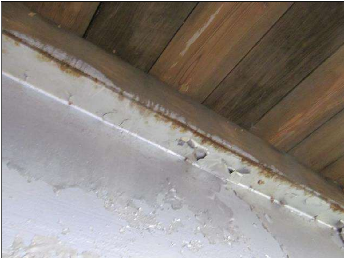
Span 1 Beam 2: SURFACE RUST SCATTERED THROUGH OUT TOP AND BOTTOM FLANGES. NO LOSS OF SECTION
