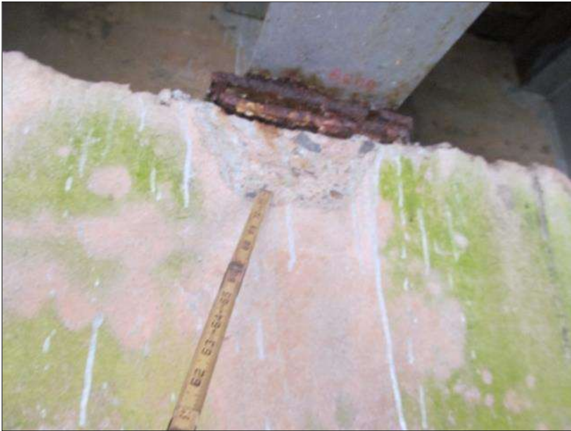
Bent 1 Abutment: 1" DEEP X 5" ROUND AREA OF SPALLING UNDER BEAM 6
