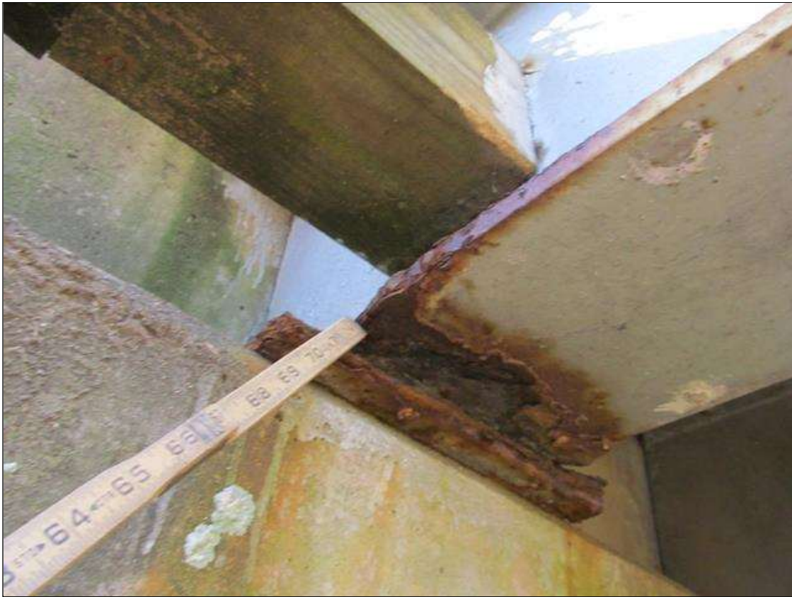
Span 1 Beam 10: SECTION LOSS TO BOTTOM FLANGE AT ABUTMENT 2, REMAINING THICKNESS IS .0104 DOWN TO KNIFE EDGE, PAR ISSUED
