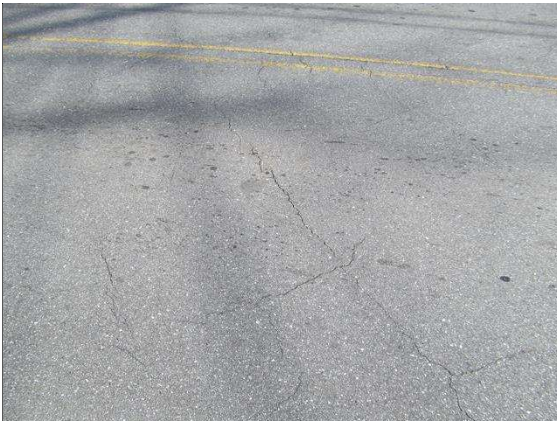
Span 1 Wearing Surface: SCATTERED CRACKING THROUGH OUT WEARING SURFACE. CRACKING IS UP TO .0104.
