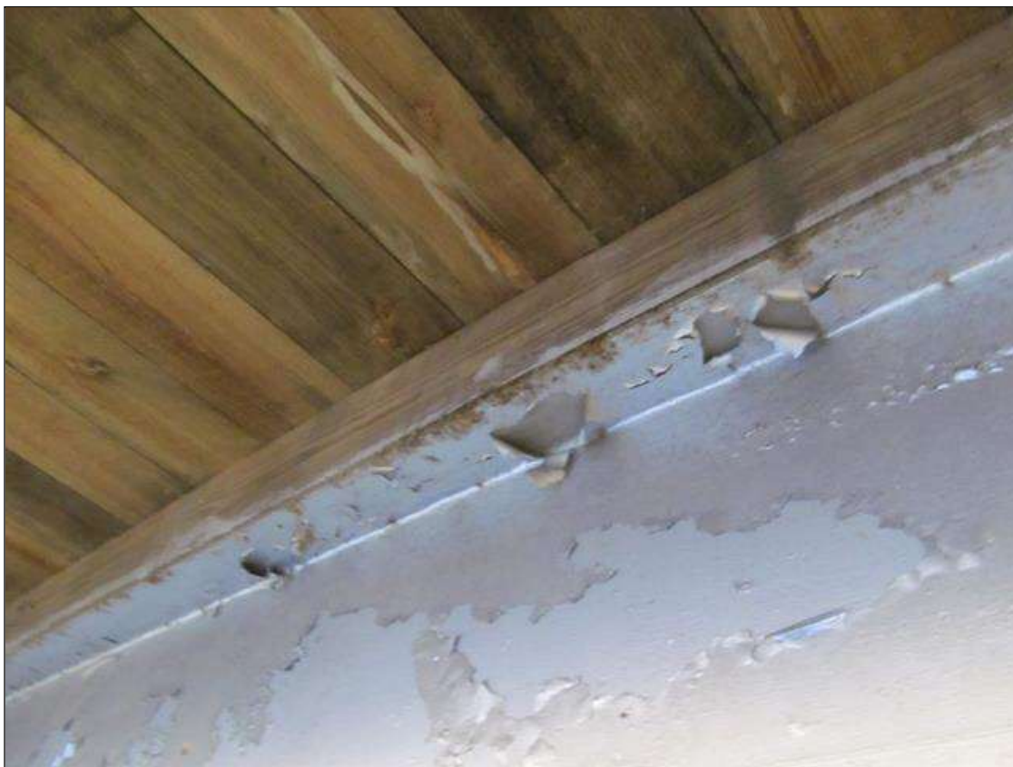
Span 1 Beam 7: SURFACE RUST SCATTERED THROUGH OUT TOP AND BOTTOM FLANGES. NO LOSS OF SECTION
