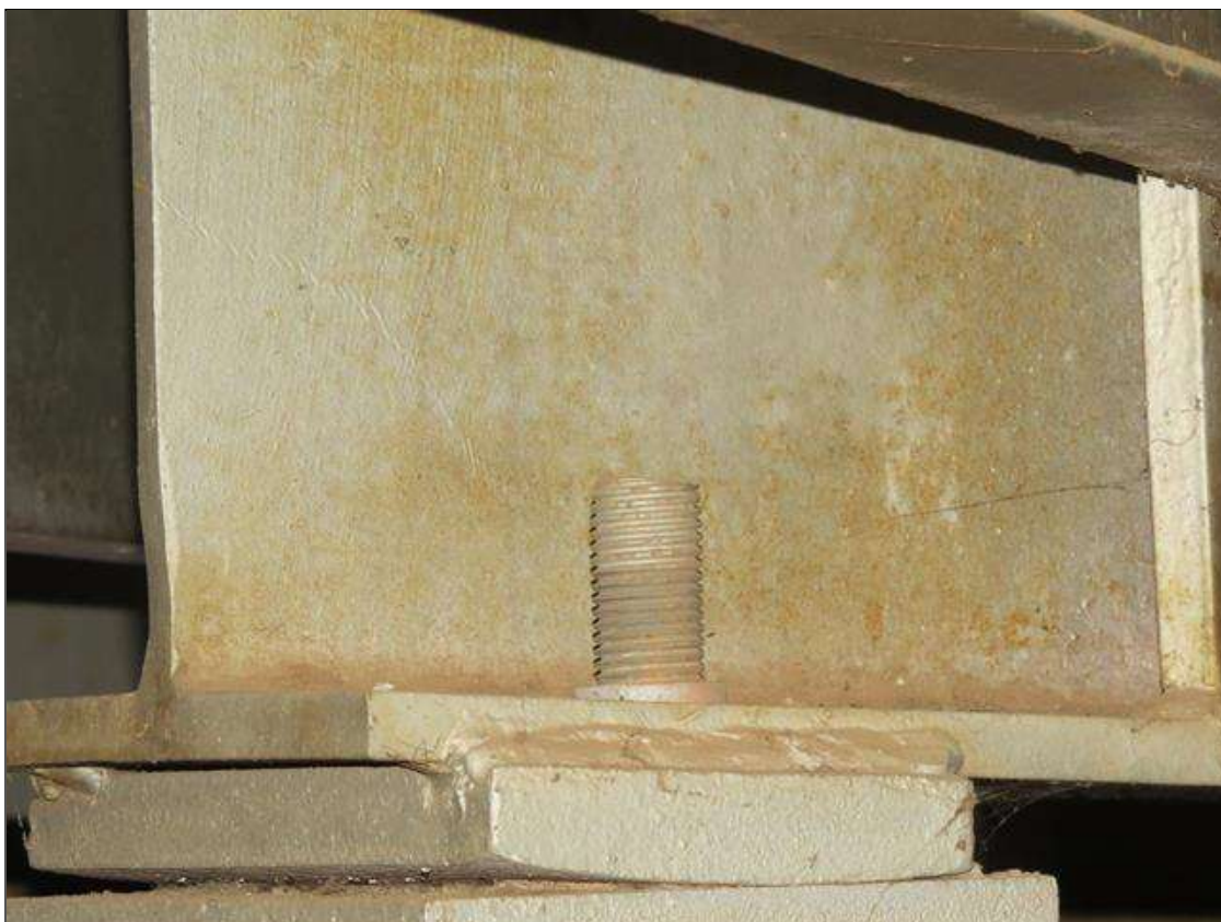
SPAN 1 BEAM 5 FAR BEARING - LEFT SIDE ANCHOR NUT MISSING (PAR PHOTO)
