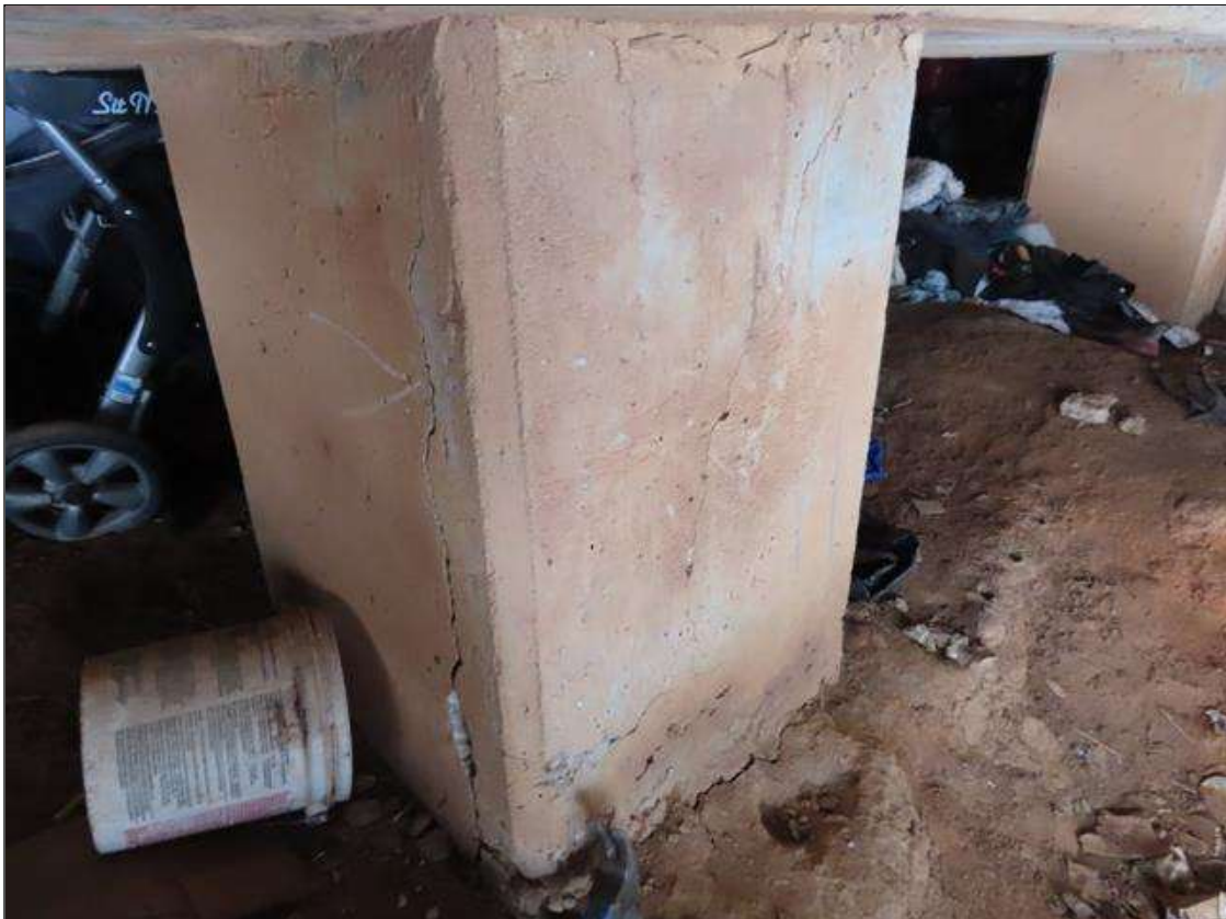
TYP. VERTICAL 1/4IN CRACKING & DELAMINATION (UP TO FULL WIDTH X 3FT H.) THROUGHOUT FAR FACE OF BENT 1 COLUMNS, COLUMN 11
