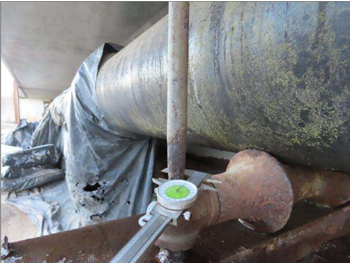
SPAN 1 RIGHT OVERHANG UTILITY - SECTION LOSS (1/4IN SL, 5/8IN REMAIN) TO BOTH HANGERS AT FAR END (PAR PHOTO)
