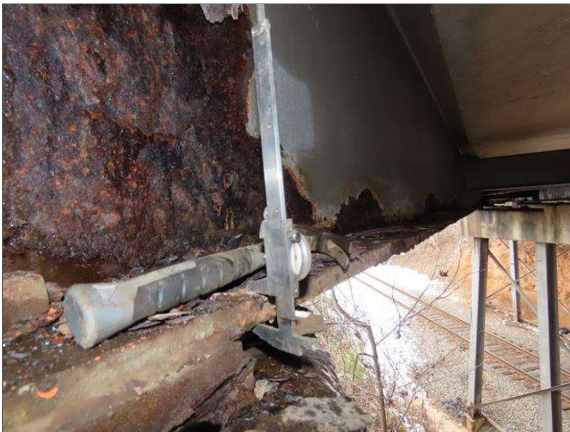
SPAN 4 BEAM 11 - BOTTOM FLANGE SECTION LOSS (UP TO 36% SL, 5/16IN SL, 9/16IN REMAIN) TO FULL WIDTH FOR 15FT L. & WEB SECTION LOSS (1/8IN SL, 7/16IN REMAIN) X 5IN H. FOR 15FT L. AT FAR END (PAR PHOTO)
