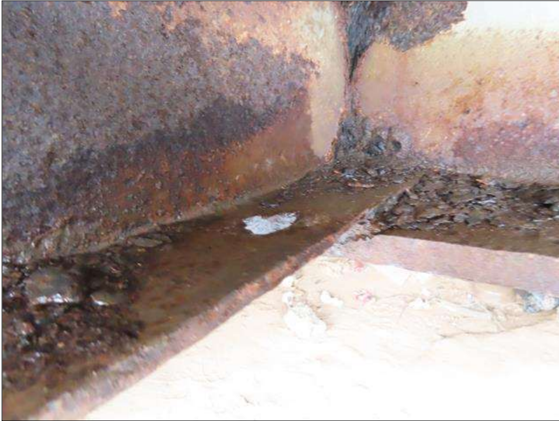
SPAN 1 RIGHT OVERHANG UTILITY - BRACKET SECTION LOSS (UP TO 100%, AVG. 3/16IN REMAIN) AT CONNECTION TO BEAM 11 BOTTOM FLANGE AT FAR END (PAR PHOTO)
