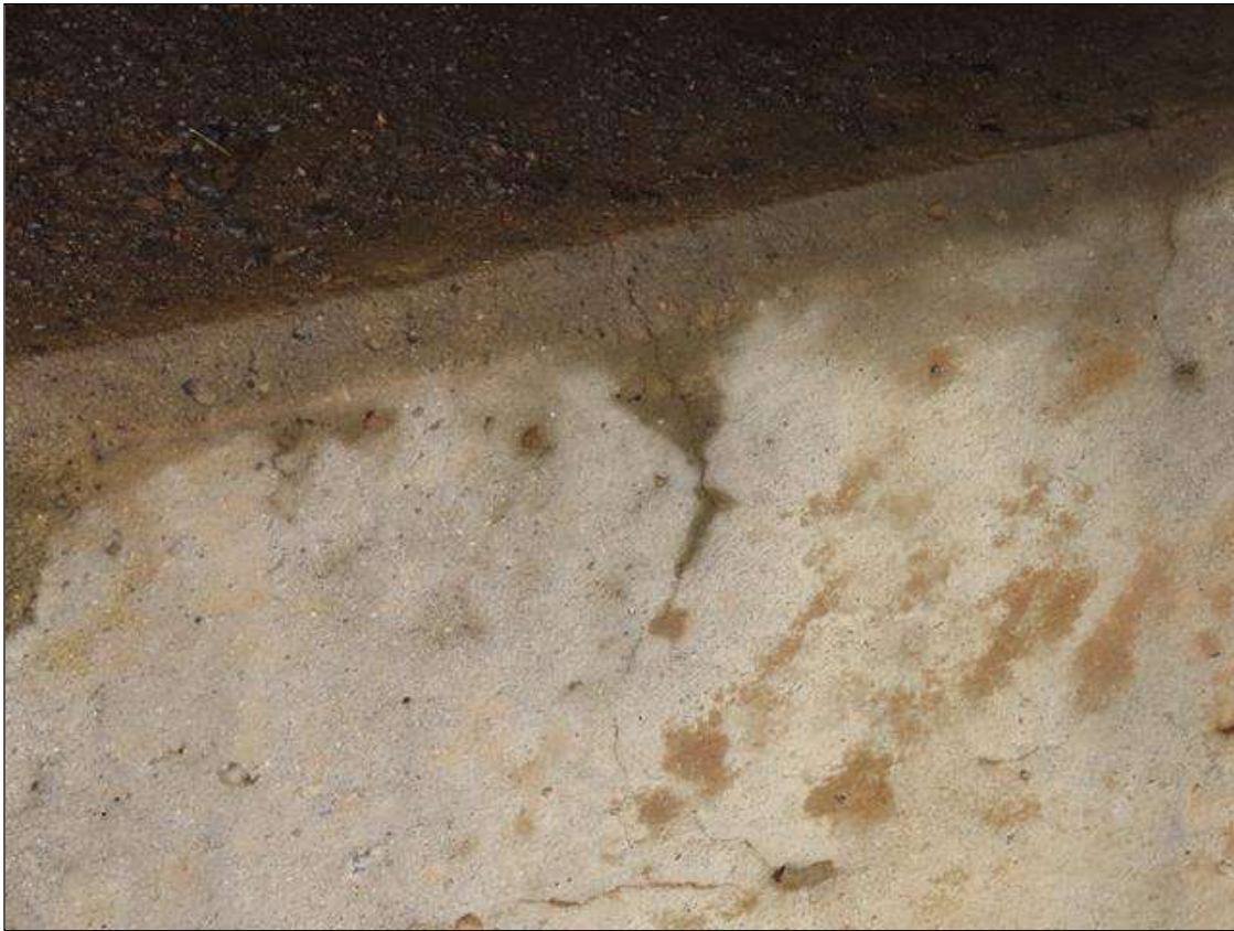
TYP. INTERMITTENT VERTICAL HAIRLINE CRACKING (UP TO FULL HEIGHT) THROUGHOUT END BENT 1 CAP, BELOW BAY 10
