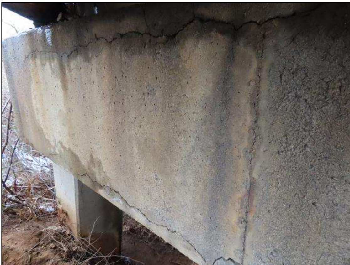
BENT 4 CAP - DELAMINATION (FULL HEIGHT) & 2X SPALLS (UP TO 48IN X 16IN X 3IN) WITH EXPOSED REBAR TO FAR FACE BELOW BAYS 8-10 (25FT TOTAL) (PAR PHOTO 1/3)
