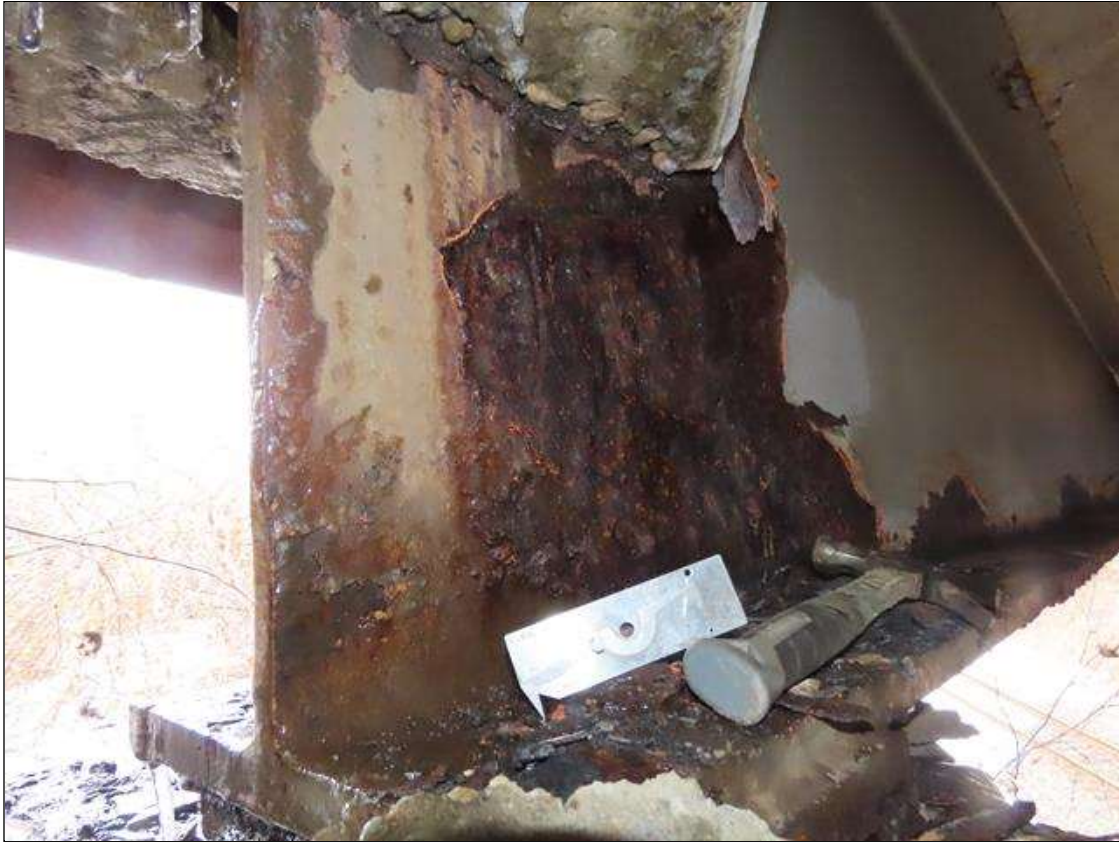
SPAN 4 BEAM 11- WEB SECTION LOSS (1/8IN SL, 7/16IN REMAIN) FOR 20IN L. X 20IN H. AT FAR END DIAPHRAGM
