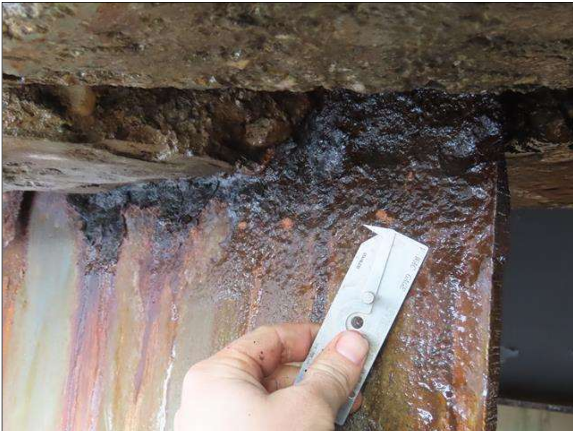
SPAN 3 BEAM 11 - WEB SECTION LOSS (7/16IN SL, 1/8IN REMAIN) FOR 18IN L. X 4IN H. AT FAR END DIAPHRAGM (PAR PHOTO)
