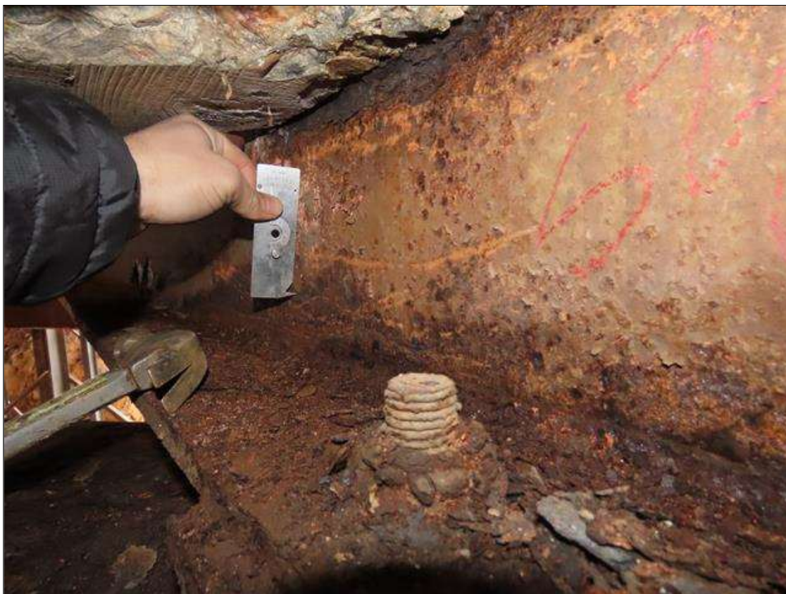
SPAN 2 BEAM 9 - WEB SECTION LOSS (1/16IN SL, 7/16IN REMAIN) TO BOTTOM FOR 24IN L. X 3IN H. AT NEAR END
