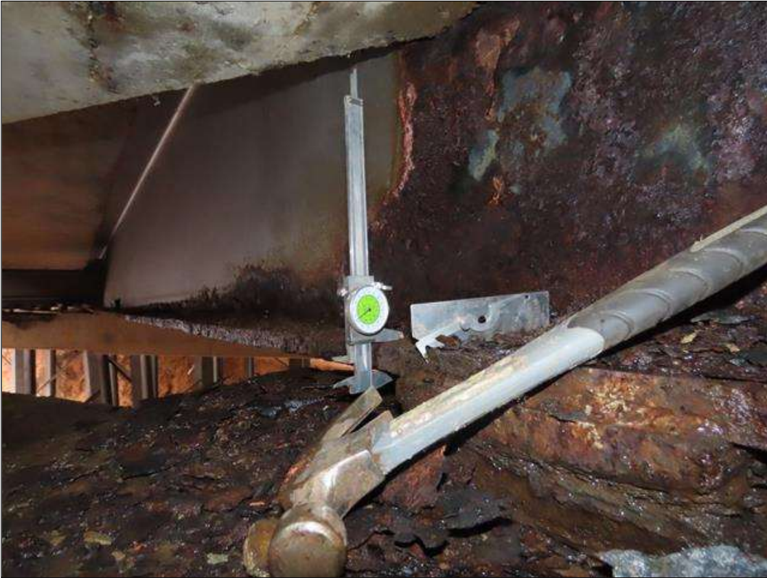
SPAN 4 BEAM 7 - BOTTOM FLANGE SECTION LOSS (UP TO 22% SL, 3/16IN SL, 11/16IN REMAIN) TO FULL WIDTH FOR 12FT & WEB SECTION LOSS (1/8IN SL, 7/16IN REMAIN) X 5IN H. FOR 1/2 L. AT FAR END
