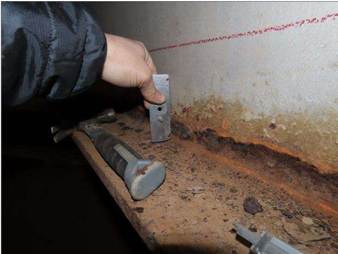
SPAN 1 BEAM 7 - WEB SECTION LOSS (3/16IN SL, 5/16IN REMAIN) TO RIGHT SIDE, 2IN H. FOR 6FT L. STARTING 10FT FROM FAR END (PAR PHOTO)
