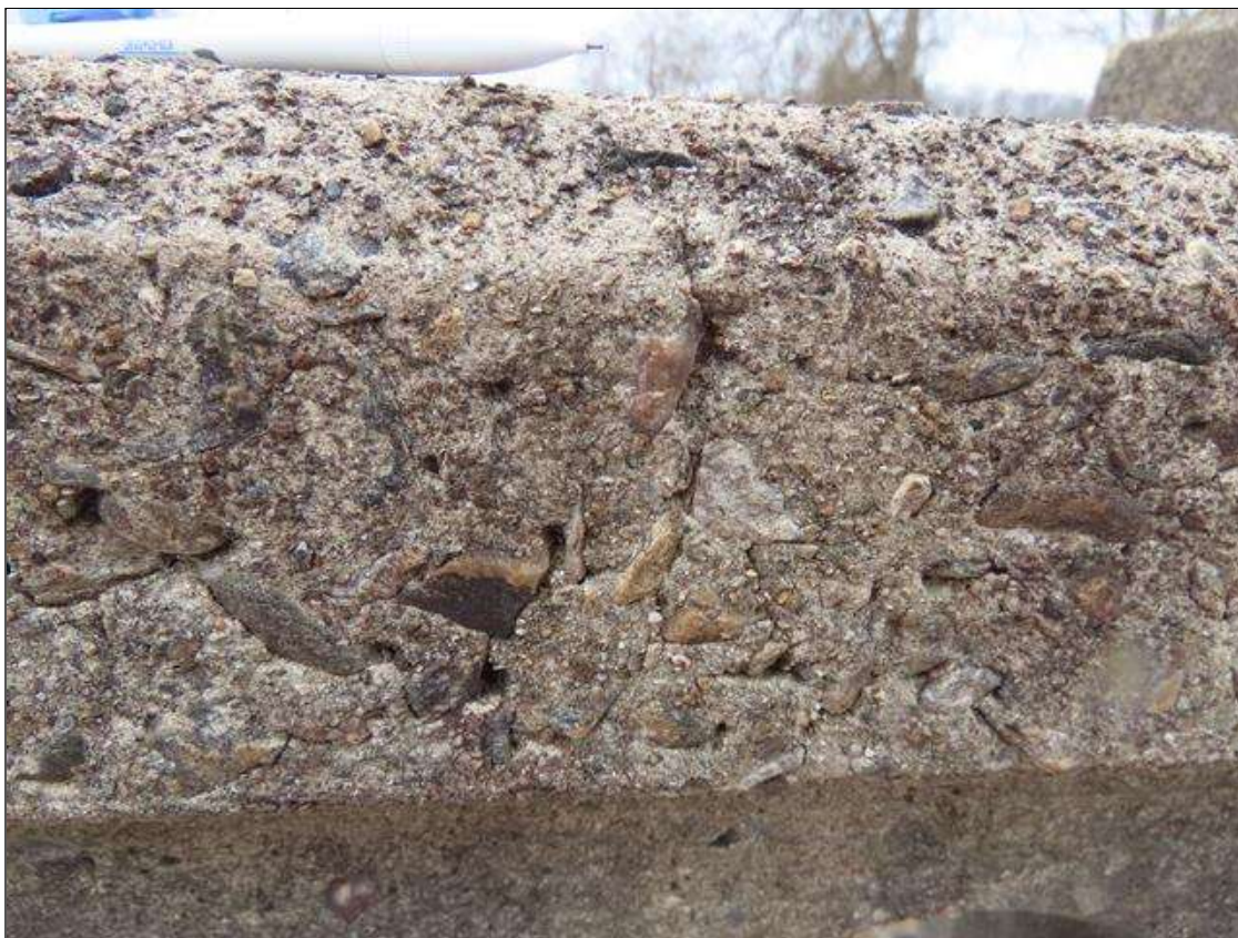
TYP. INTERMITTENT 1/32IN VERTICAL CRACKING THROUGHOUT RAILS, SPAN 1 RIGHT RAIL
