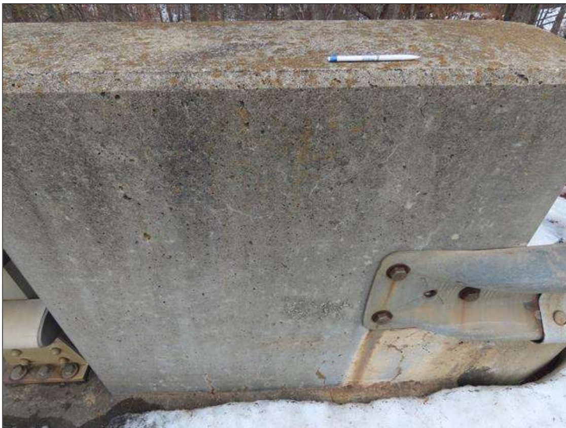
SPAN 5 LEFT RAIL - HAIRLINE MAP CRACKING (5 SQ. FT.) THROUGHOUT CONCRETE END POST
