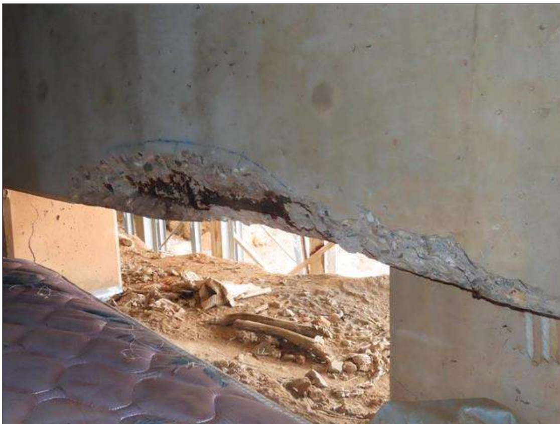
BENT 1 CAP - SPALL (48IN X 12IN X 5IN) WITH EXPOSED REBAR TO NEAR BOTTOM CORNER BELOW BAY 9 (PAR PHOTO)
