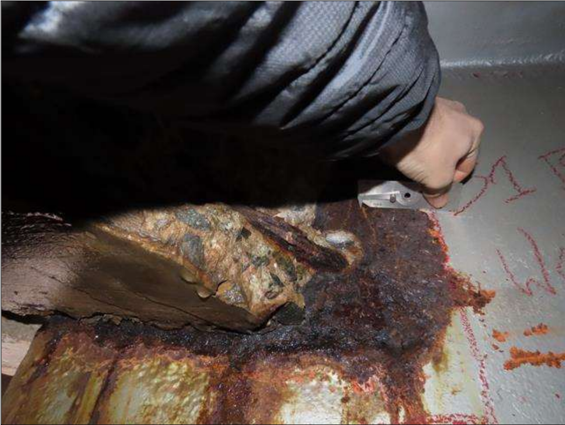
SPAN 1 BEAM 8 - WEB SECTION LOSS (1/4IN SL, 1/4IN REMAIN) FOR 16IN L. X 8IN H. AT FAR END DIAPHRAGM (PAR PHOTO)
