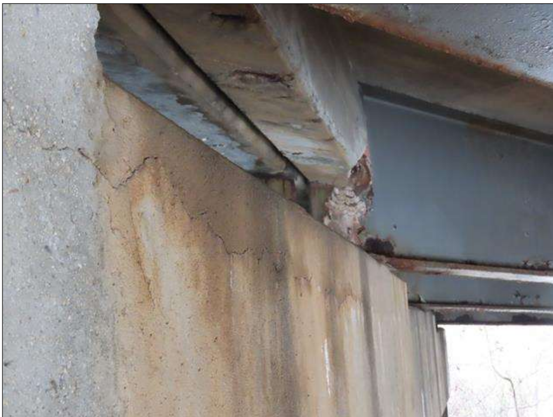
BENT 4 CAP - HORIZONTAL 1/8IN CRACKING & DELAM (UP TO 8IN H.) FOR 25FT BELOW BAYS 7-9
