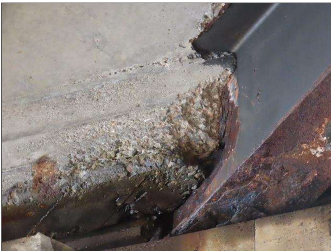
SPAN 3 BAY 7 NEAR DIAPHRAGM - SPALL (16IN X 16IN X 5IN) WITH EXPOSED REBAR ADJACENT TO BEAM 7 (PAR PHOTO)
