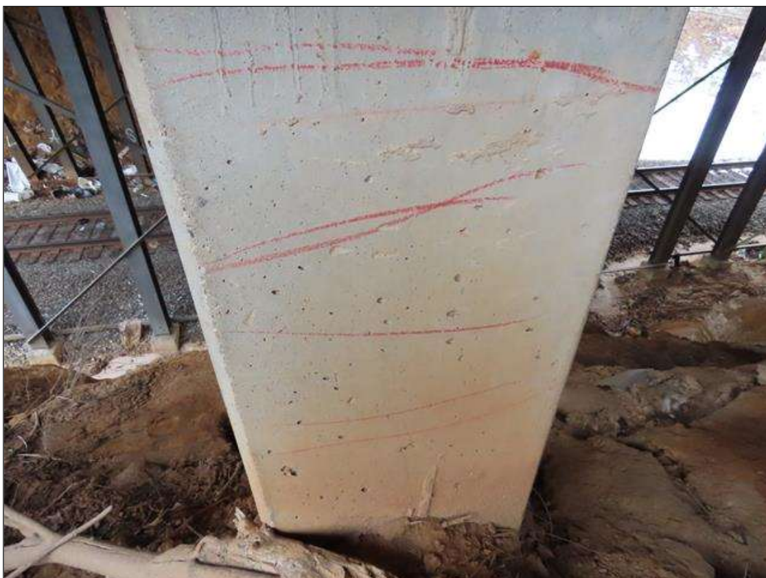
BENT 4 COLUMN 16 - DELAMINATION (3FT H. X FULL WIDTH) TO FAR FACE (COLUMN 15, 17 SIMILAR)
