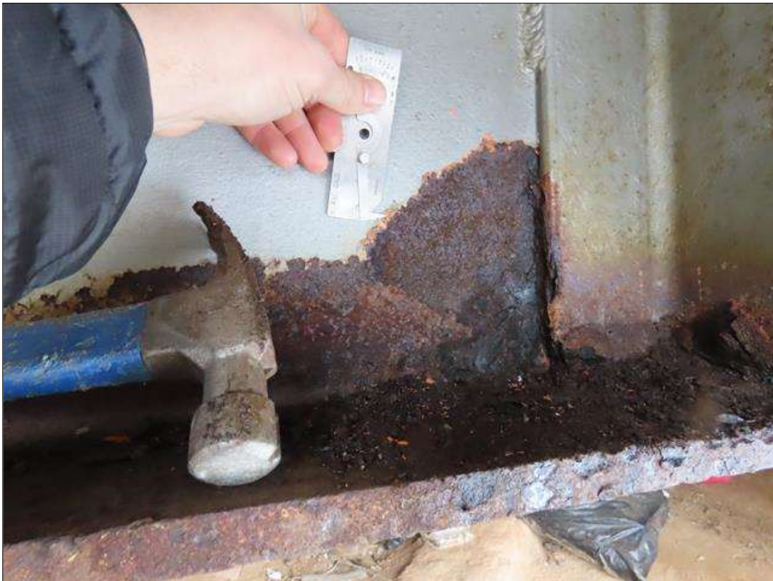
SPAN 1 BEAM 11 - WEB SECTION LOSS (3/16IN PITTING, 5/16IN REMAIN) TO RIGHT SIDE, 6IN X 6IN AT BOTH SIDES OF UTILITY BRACKET CONNECTION, 6FT FROM FAR END (PAR PHOTO)
