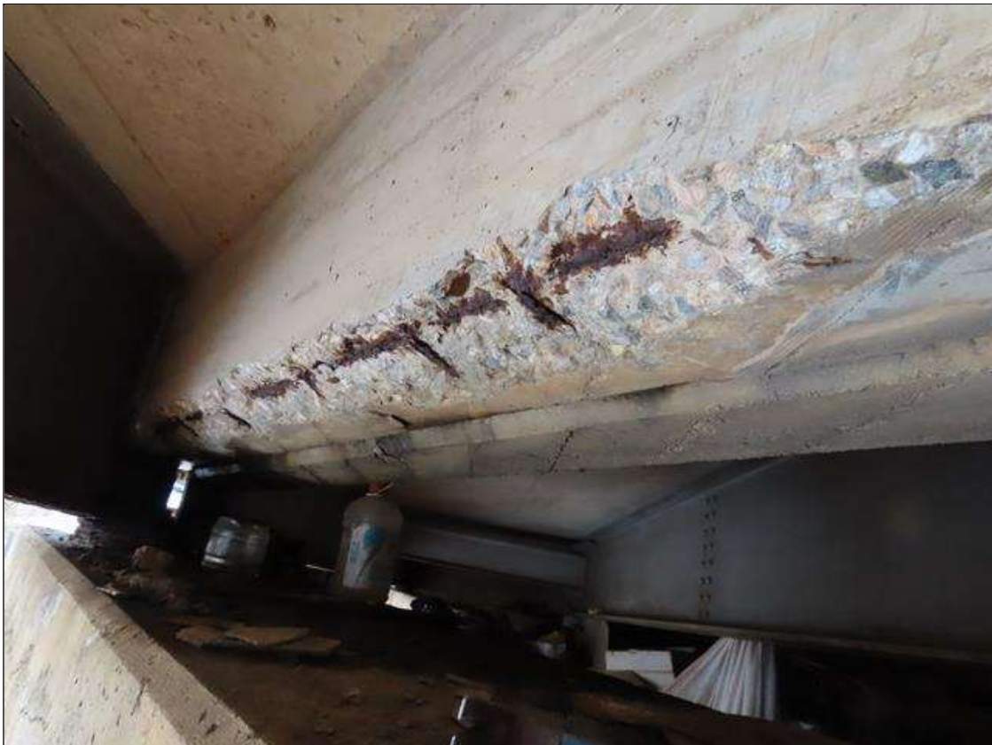
SPAN 2 BAY 10 NEAR DIAPHRAGM - SPALL (6FT X 7IN X 3IN) WITH EXPOSED REBAR THROUGHOUT (PAR PHOTO)
