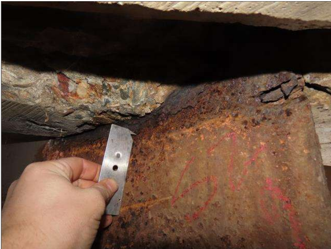
SPAN 2 BEAM 9 - WEB SECTION LOSS (UP TO 100% SL, AVG. 1/8IN REMAIN) FOR 20IN L. X 2IN H. AT NEAR END DIAPHRAGM (PAR PHOTO)
