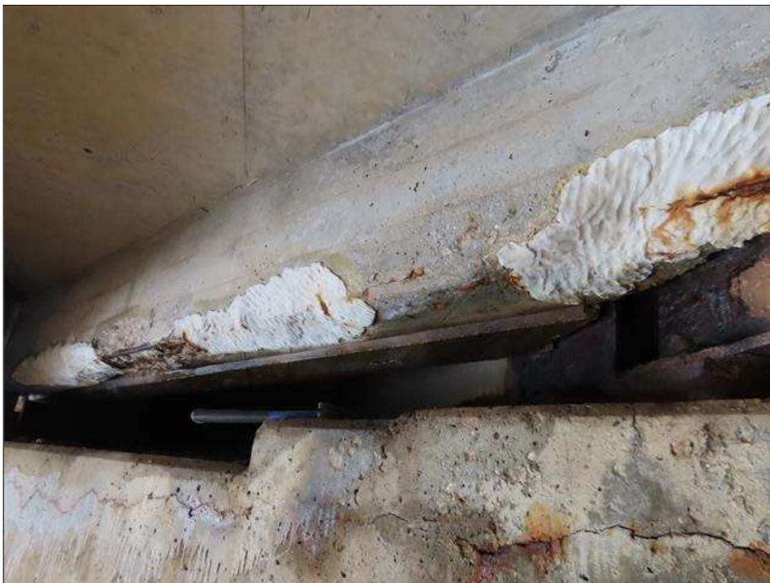
SPAN 2 BAY 7 NEAR DIAPHRAGM - FAILED REPAIR WITH SPALLING (UP TO 30IN X 12IN X 6IN) WITH EXPOSED REBAR THROUGHOUT (PAR PHOTO)
