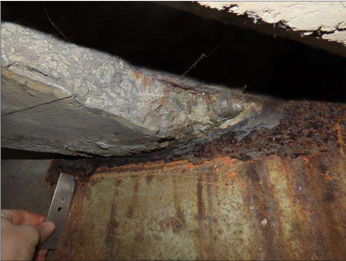
SPAN 2 BEAM 10 - WEB SECTION LOSS (5/16IN SL, 3/16IN REMAIN) FOR 18IN L. X 3IN H. AT NEAR END DIAPHRAGM (PAR PHOTO)
