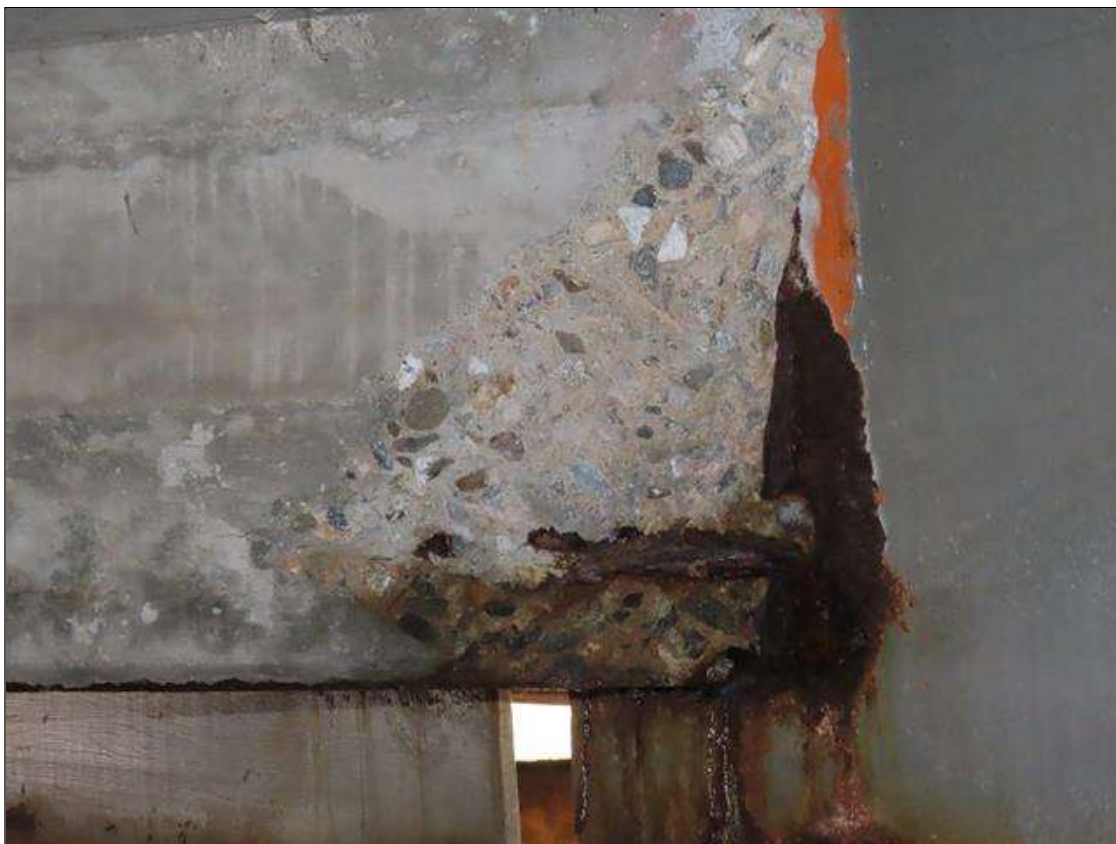
SPAN 1 BAY 7 FAR DIAPHRAGM - SPALL (18IN X 16IN X 3IN) WITH EXPOSED REBAR ADJACENT TO BEAM 8 (PAR PHOTO)
