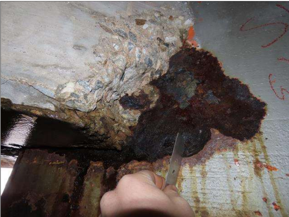
SPAN 1 BEAM 11 - WEB SECTION LOSS (3/8IN SL, 1/8IN REMAIN) FOR 18IN L. X 9IN H. AT FAR END DIAPHRAGM (PAR PHOTO)
