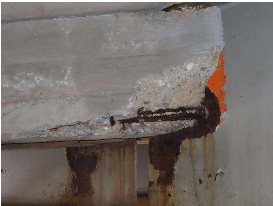
SPAN 5 BAY 9 NEAR DIAPHRAGM - SPALL (26IN X 12IN X 4IN) WITH EXPOSED REBAR ADJACENT TO BEAM 9 (PAR PHOTO)
