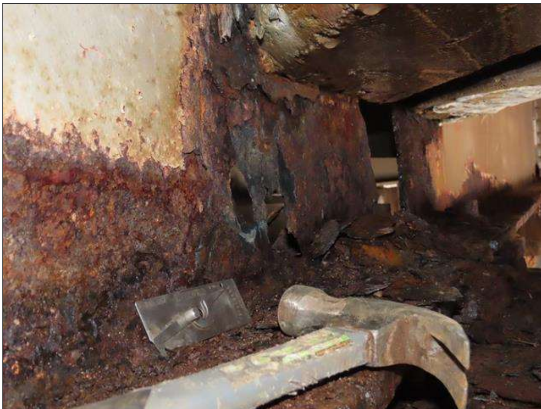
SPAN 1 BEAM 7 - WEB SECTION LOSS (UP TO 100% SL, AVG. 1/8IN REMAIN) FOR 16IN L. X 8IN H. AT FAR END DIAPHRAGM (PAR PHOTO)
