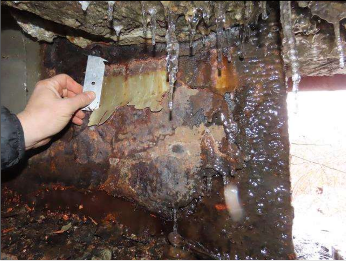
SPAN 5 BEAM 11 - WEB SECTION LOSS (UP TO 1/2IN SL, 5/16IN REMAIN) FOR 20IN L. X 20IN H. AT NEAR END DIAPHRAGM (PAR PHOTO)
