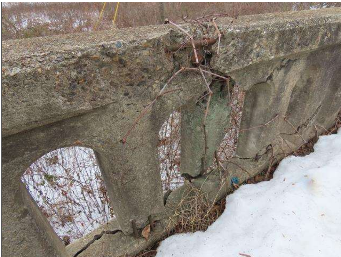
SPAN 5 RIGHT RAIL - HEAVY IMPACT DAMAGE (FULL HEIGHT X 10FT L.) WITH BROKEN/SPALLED CONCRETE & EXPOSED REBAR STARTING 5FT FROM NEAR END (PAR PHOTO 2/2)
