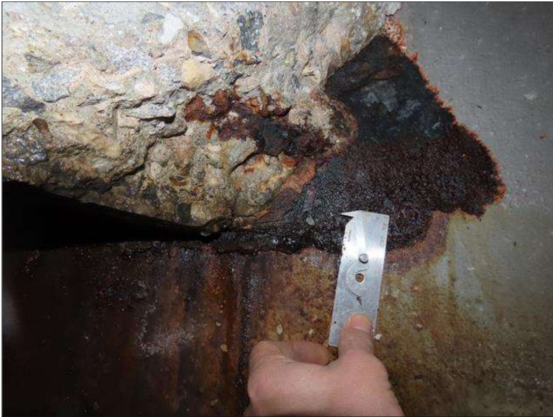
SPAN 2 BEAM 11 - WEB SECTION LOSS (UP TO 7/16IN SL, AVG. 1/8IN REMAIN) FOR 12IN L. X 6IN H. AT FAR END DIAPHRAGM (PAR PHOTO)
