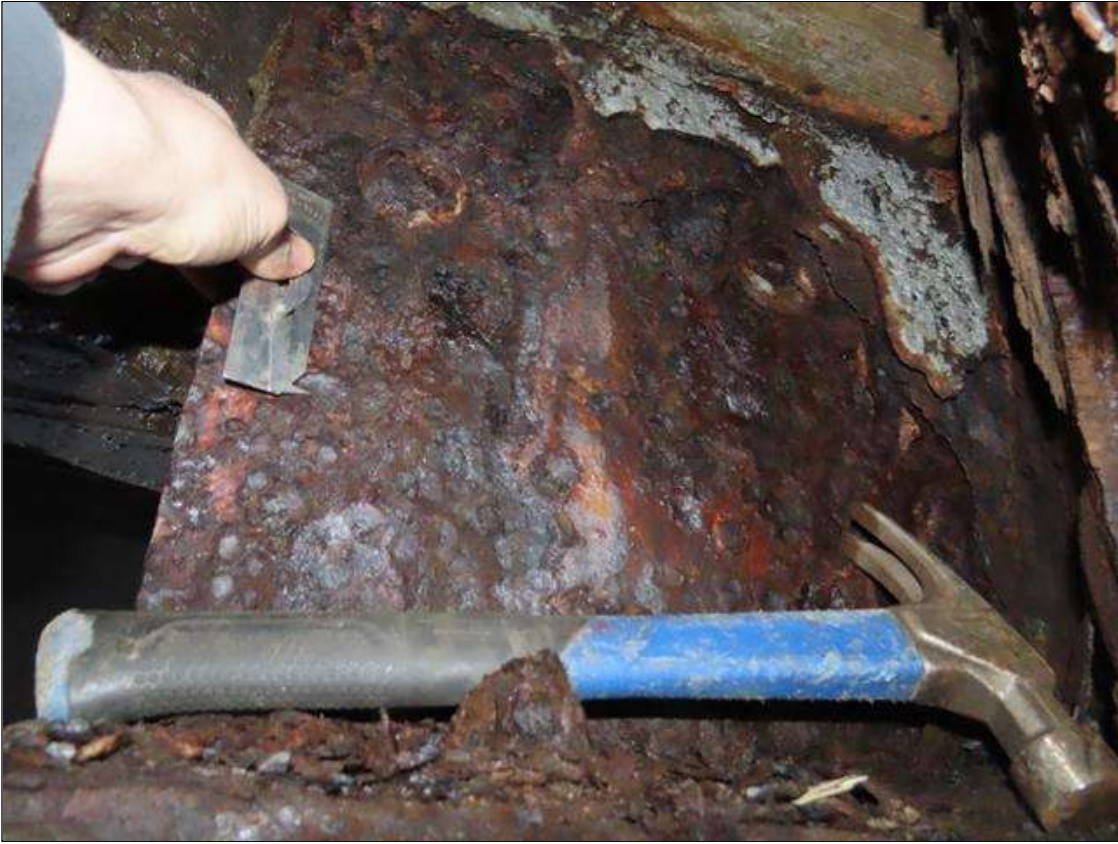
SPAN 2 BEAM 7 - WEB SECTION LOSS (UP TO 100% SL, AVG. 3/16IN REMAIN) TO FULL HEIGHT FOR 18IN L. AT FAR END DIAPHRAGM (PAR PHOTO)
