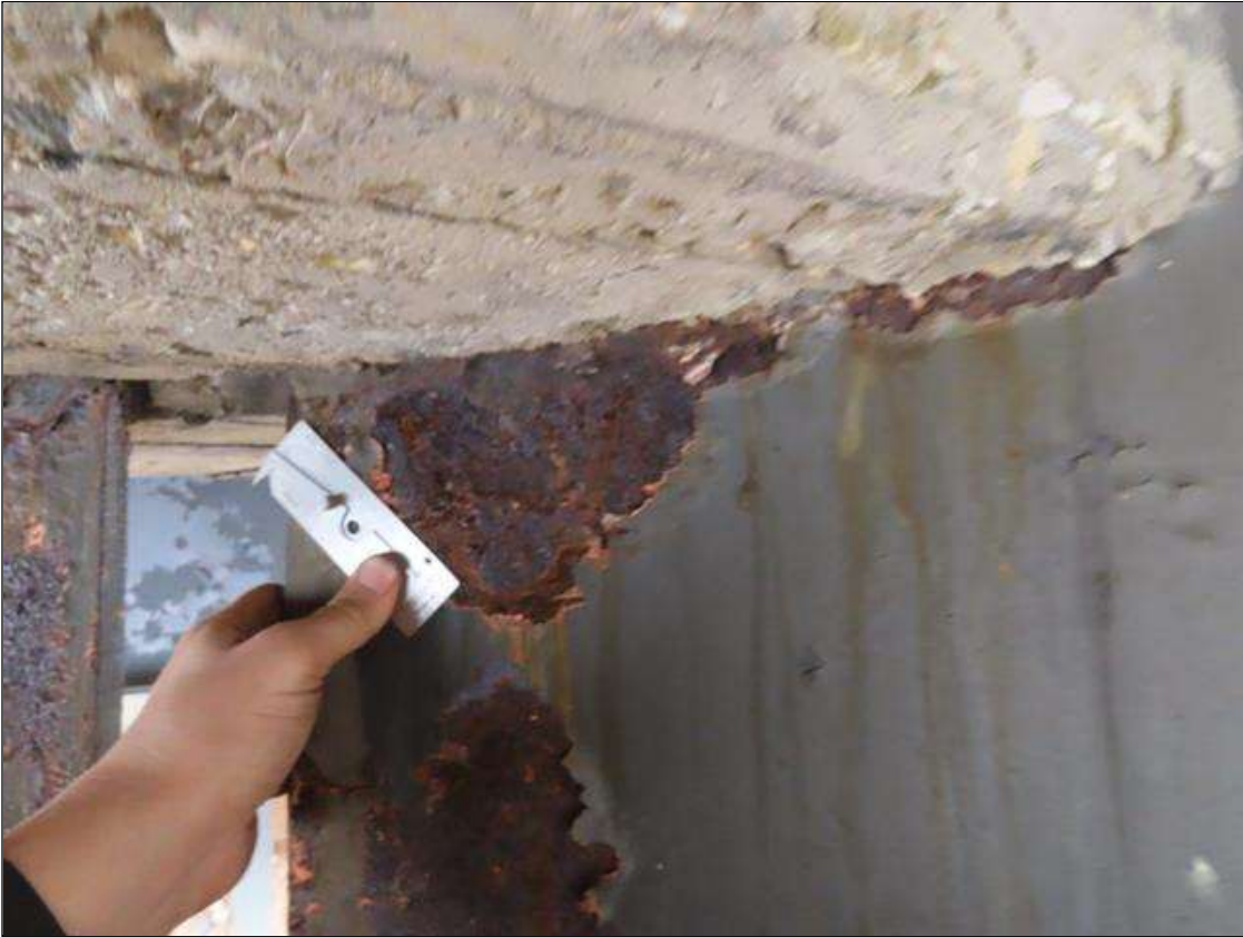
SPAN 4 BEAM 9 - WEB SECTION LOSS (3/8IN SL, 1/4IN REMAIN) FOR 6IN L. X 3IN H. AT NEAR END DIAPHRAGM (PAR PHOTO)
