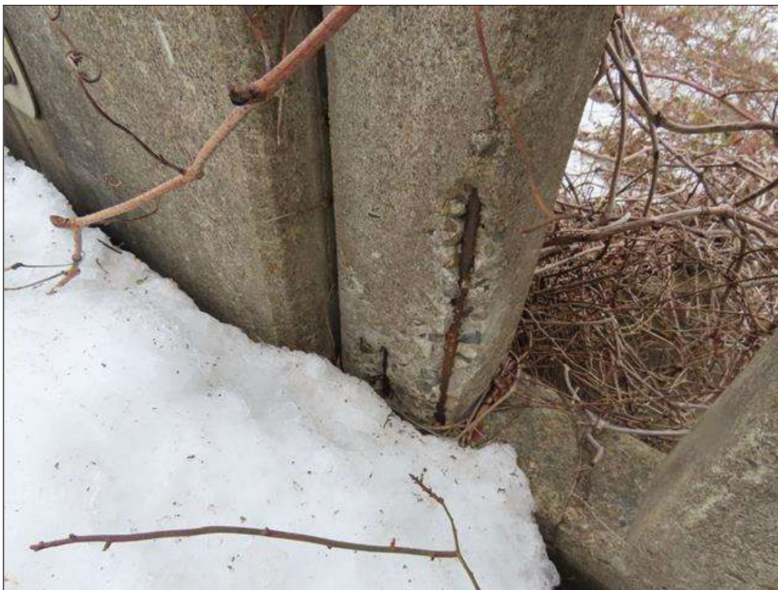
SPAN 5 RIGHT RAIL - SPALL (12IN X 5IN X 1IN) WITH EXPOSED REBAR TO NEAR SIDE OF FAR VERTICAL POST
