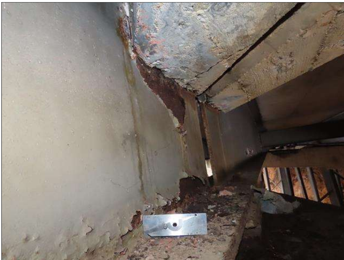
SPAN 5 BEAM 8 - WEB SECTION LOSS (1/16IN SL, 9/16IN REMAIN) FOR 8IN L. X 3IN H. AT NEAR END DIAPHRAGM
