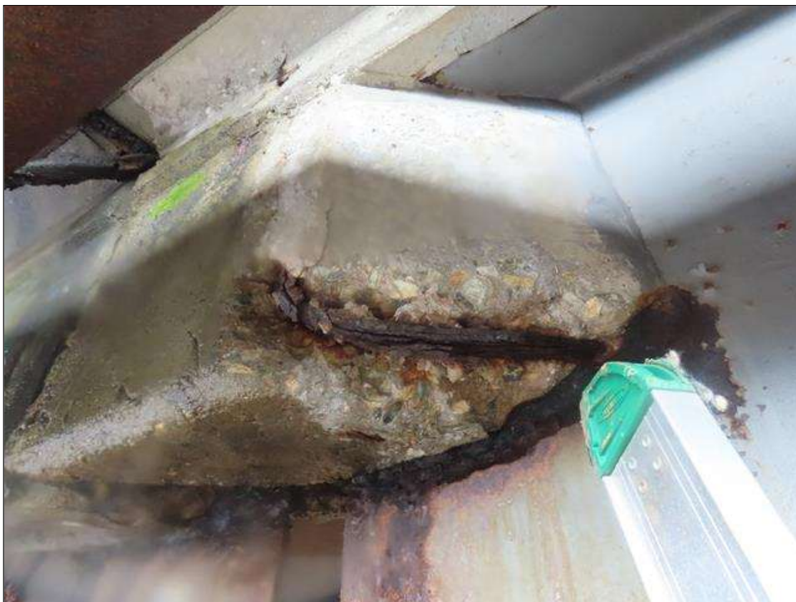
SPAN 4 RIGHT OVERHANG DIAPHRAGM AT NEAR END - SPALL (12IN X 6IN X 3IN) WITH EXPOSED REBAR (PAR PHOTO)
