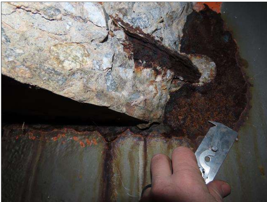
SPAN 2 BEAM 8 - WEB SECTION LOSS (UP TO 7/16IN SL, AVG. 1/8IN REMAIN) FOR 12IN L. X 6IN H. AT FAR END DIAPHRAGM (PAR PHOTO)
