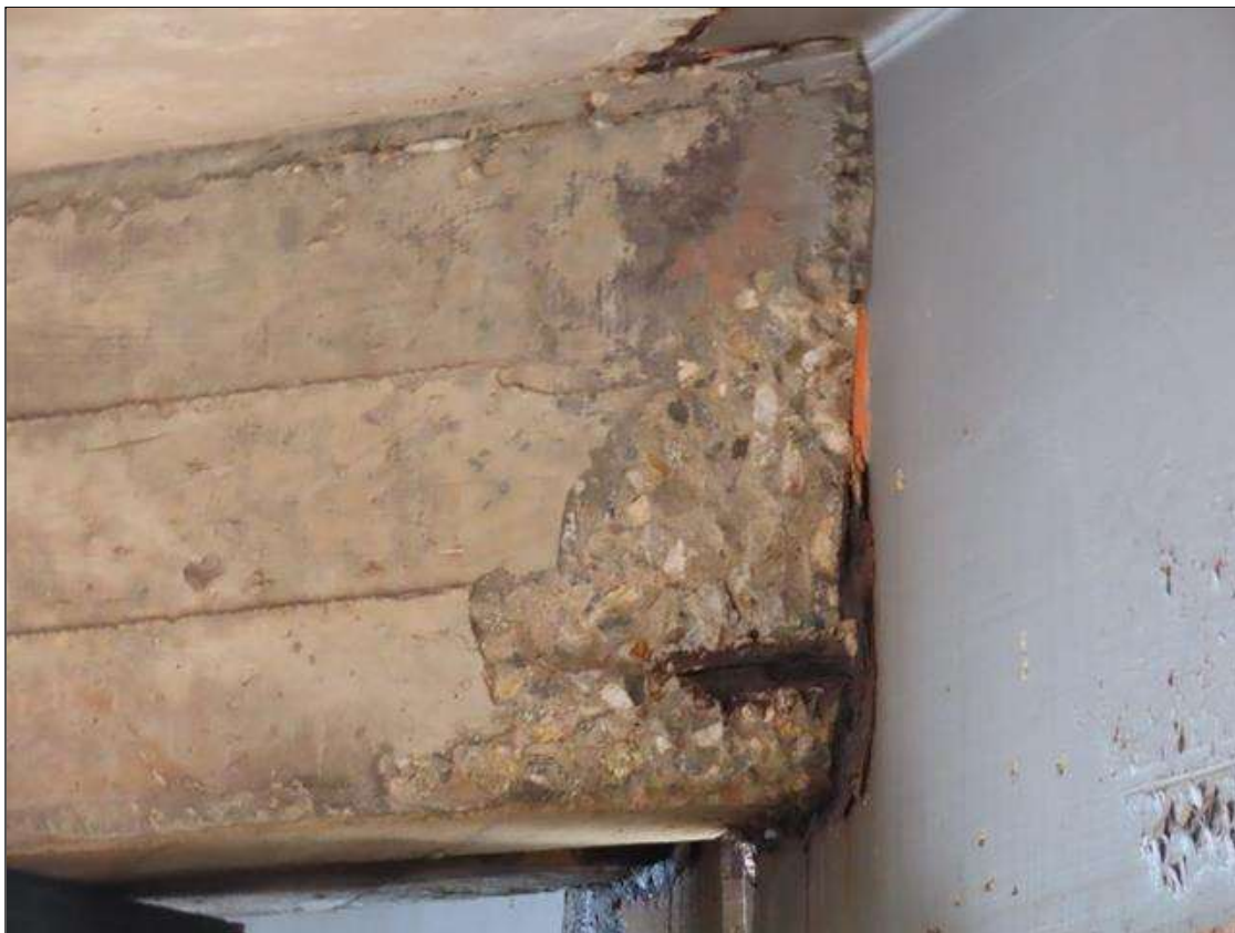
SPAN 2 BAY 7 FAR DIAPHRAGM - SPALL (12IN X 8IN X 2IN) WITH EXPOSED REBAR ADJACENT TO BEAM 8 (PAR PHOTO)
