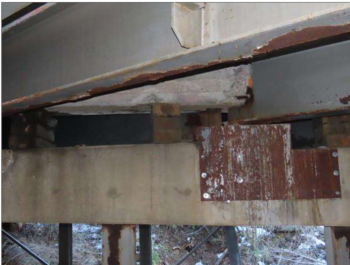
BENT 2 CAP - TIMBER CRIBBING REMAINS THROUGHOUT TOP OF CAP IN BAYS 7 & 8
