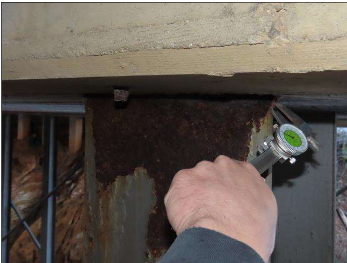
BENT 2 PILE 11 - NEAR FLANGE SECTION LOSS (1/16IN SL, 3/8IN REMAIN) TO FULL WIDTH X 3IN H. AT TOP (PILES 12, 13, 14 SIMILAR)
