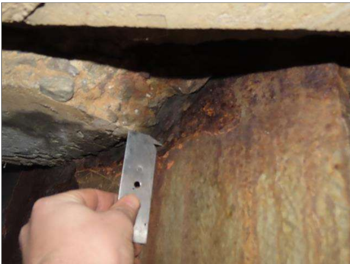
SPAN 3 BEAM 8 - WEB SECTION LOSS (UP TO 1/8IN SL, 1/2IN REMAIN) FOR 1IN W. AROUND NEAR END DIAPHRAGM
