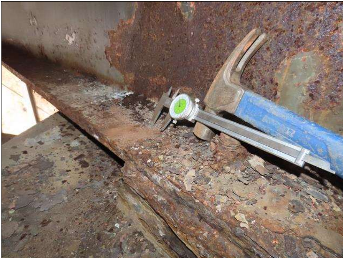
SPAN 3 BEAM 9 - BOTTOM FLANGE SECTION LOSS (UP TO 7% SL, 1/16IN SL, 7/8IN REMAIN) TO FULL WIDTH FOR 8FT L. AT FAR END
