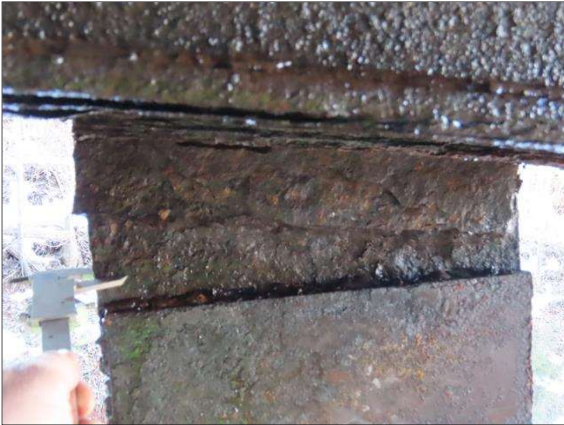
BENT 2 PILE 15 - NEAR & FAR FLANGE SECTION LOSS (UP TO 100% SL, AVG. 1/4IN REMAIN) TO FULL WIDTH, 4IN H. AT NEAR FLANGE, 4FT H. AT FAR FLANGE UNDER REAIR (PAR PHOTO 1/2)
