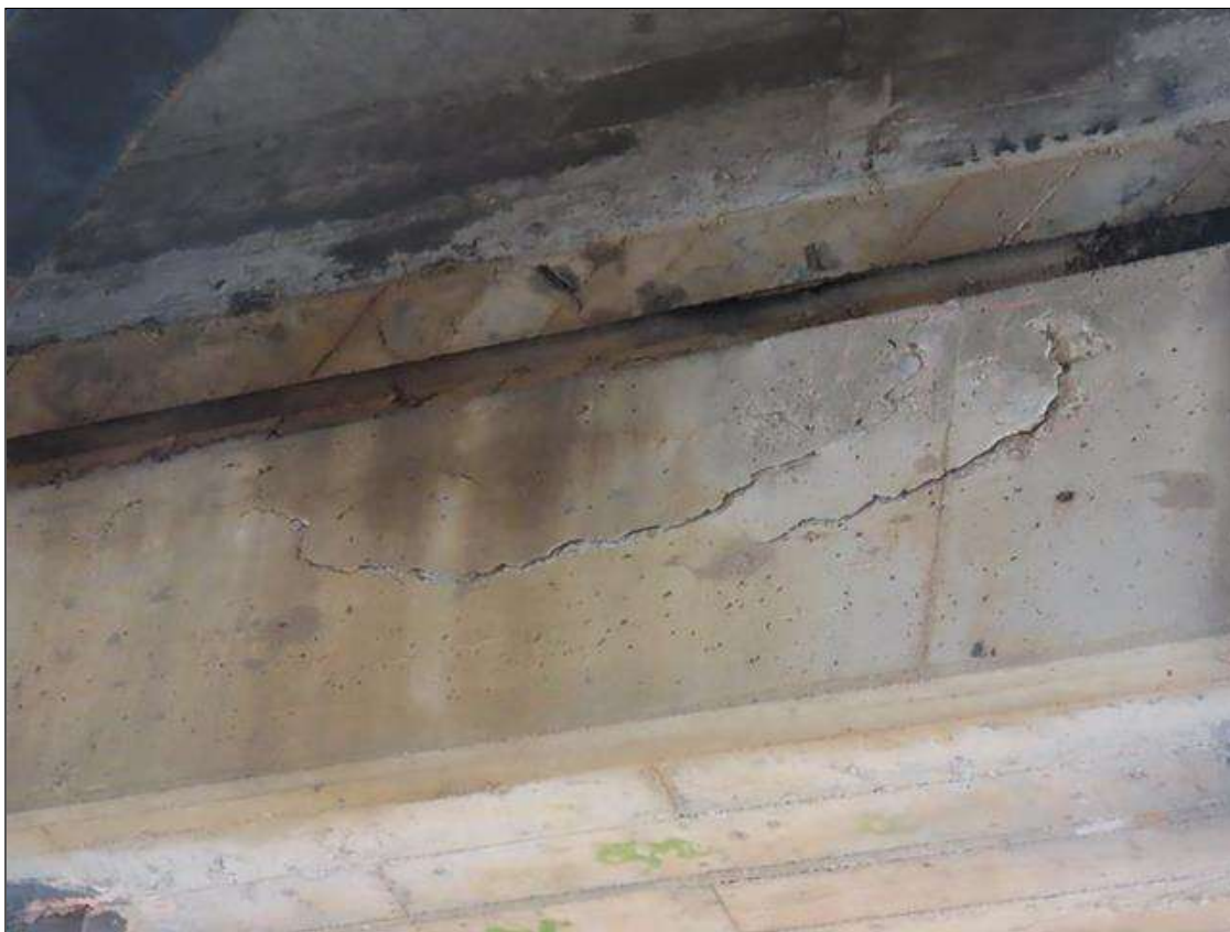
BENT 3 CAP - LOOSE DELAMINATION (4.5FT X 2FT) TO NEAR FACE BELOW BAY 8 (PAR PHOTO)
