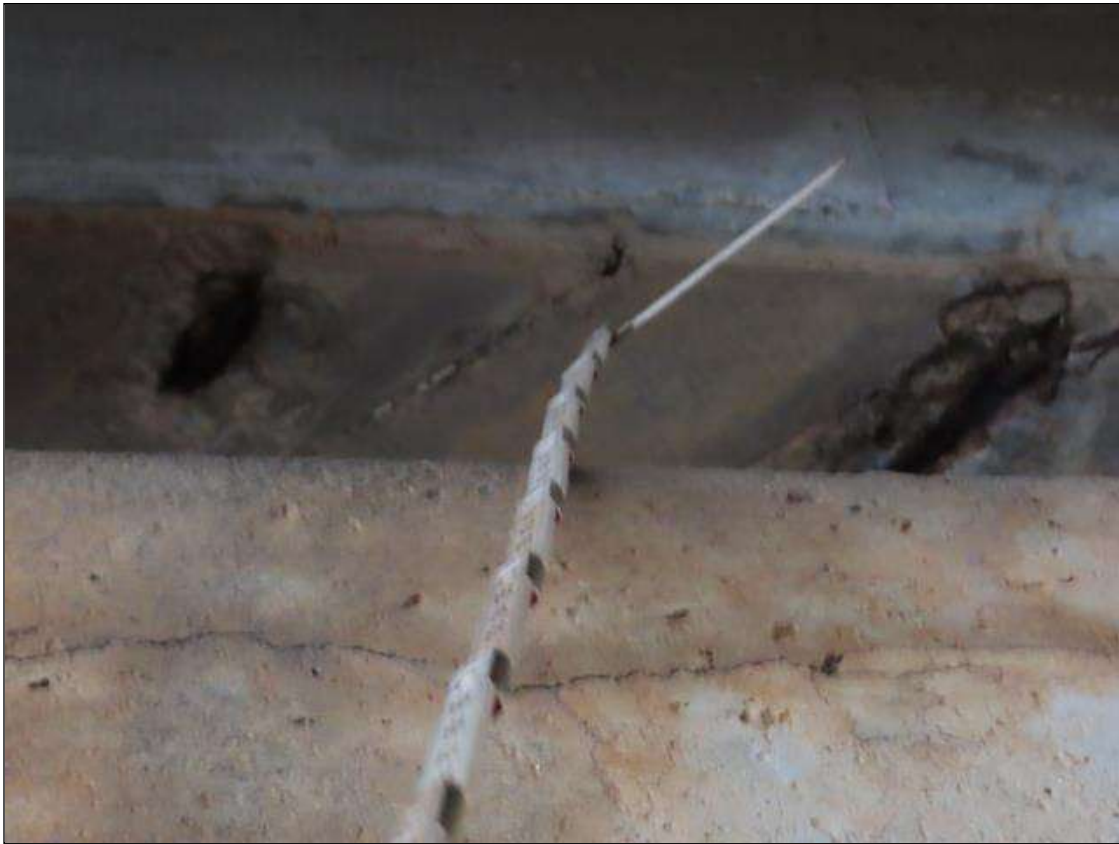
TYP. MINOR SPALLING (UP TO 8IN X 4IN X 1IN) WITH EXPOSED REBAR THROUGHOUT BOTTOM FACE OF DIAPHRAGMS, SPAN 4 BAY 7 FAR DIAPHRAGM
