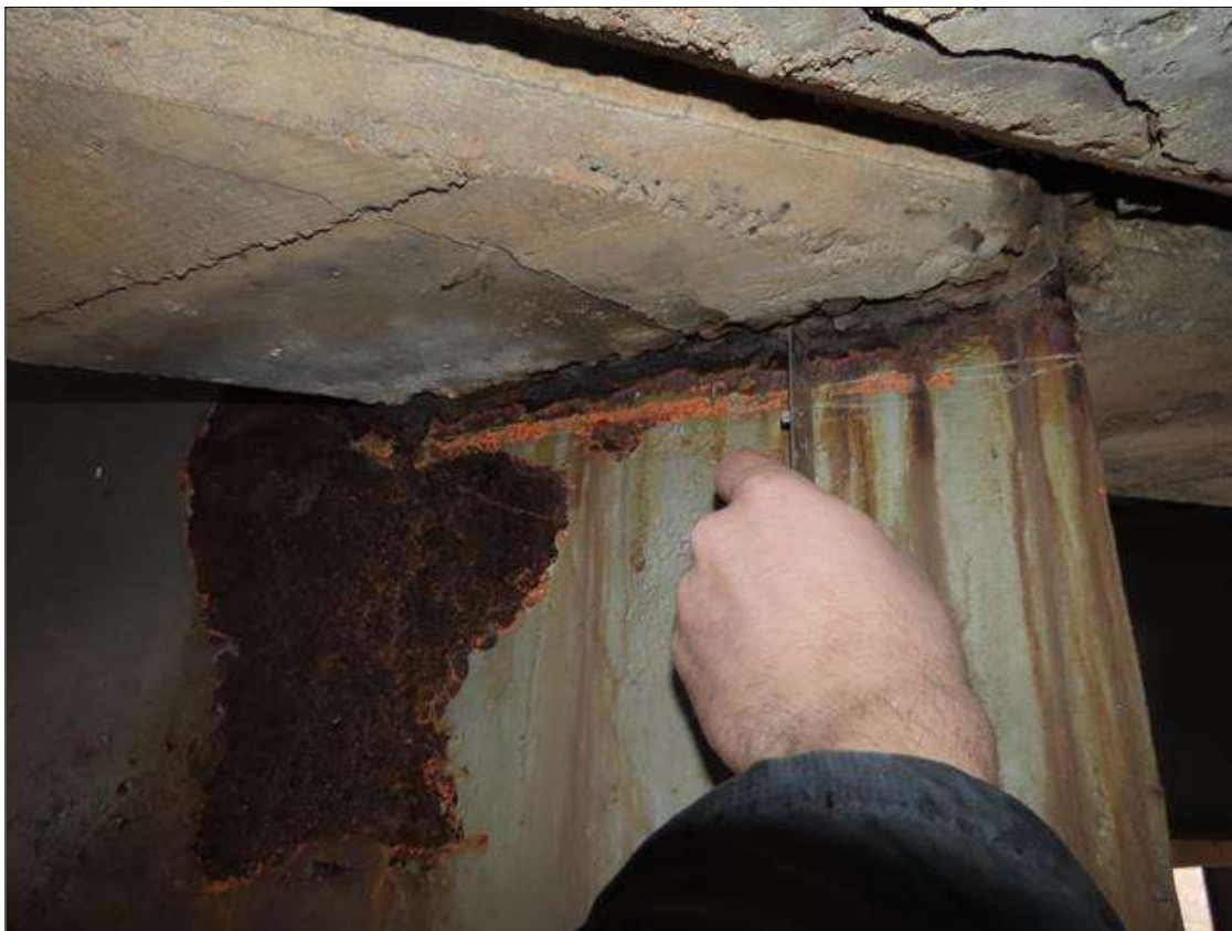
SPAN 4 BEAM 9 - WEB SECTION LOSS (1/4IN SL, 3/8IN REMAIN) FOR 20IN L. X 12IN H. AT FAR END DIAPHRAGM (PAR PHOTO)
