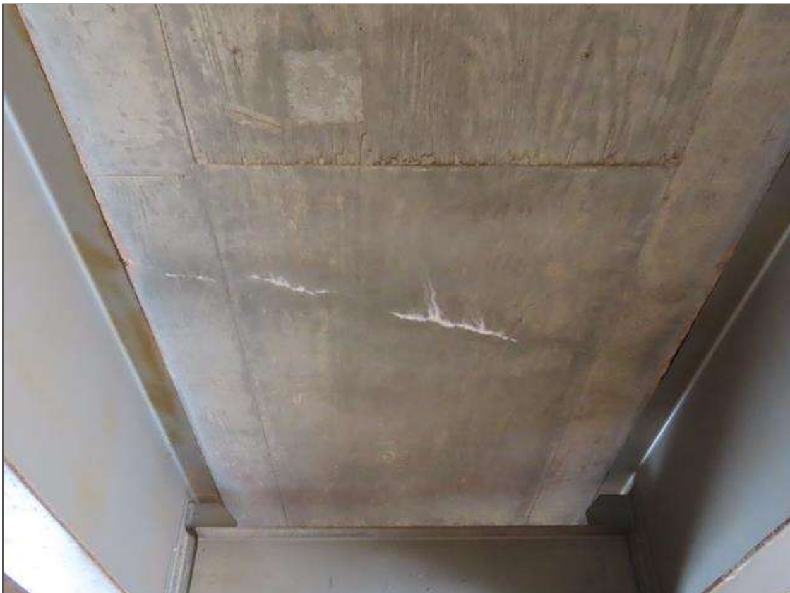
SPAN 2 DECK - TRANSVERSE HAIRLINE CRACK (8.5FT) WITH MINOR EFFLORESCENCE TO BOTTOM FACE BAY 5, 10FT FROM NEAR END
