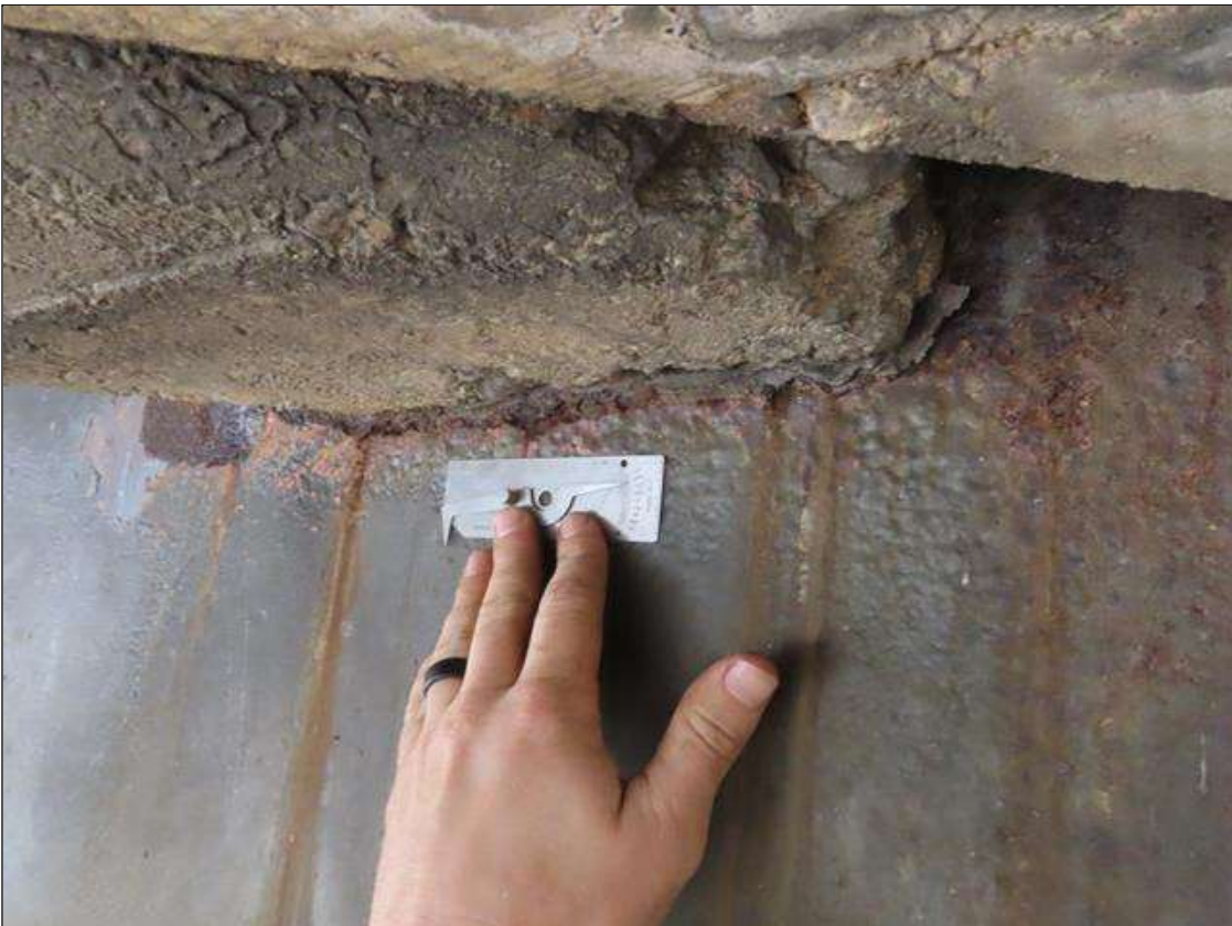
SPAN 3 BEAM 10 - WEB SECTION LOSS (1/8IN SL, 1/2IN REMAIN) FOR 12IN L. X 1IN H. AT FAR END DIAPHRAGM (SIMILAR SPAN 4 BEAM 10 AT NEAR END DIAPHRAGM)
