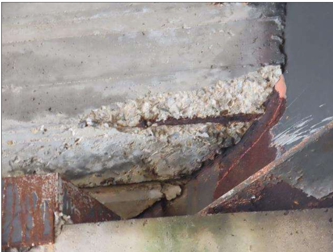
SPAN 3 BAY 8 NEAR DIAPHRAGM - SPALL (18IN X 8IN X 4IN) WITH EXPOSED REBAR ADJACENT TO BEAM 8 (PAR PHOTO)
