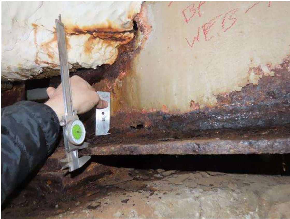
SPAN 2 BEAM 7 - BOTTOM FLANGE SECTION LOSS (UP TO 33% SL, 1/4IN SL, AVG. 1/2IN REMAIN) TO FULL WIDTH FOR 1FT L. & WEB SECTION LOSS (UP TO 100% SL, AVG. 1/8IN REMAIN) X 3IN H. FOR 5FT L. AT NEAR END (PAR PHOTO)
