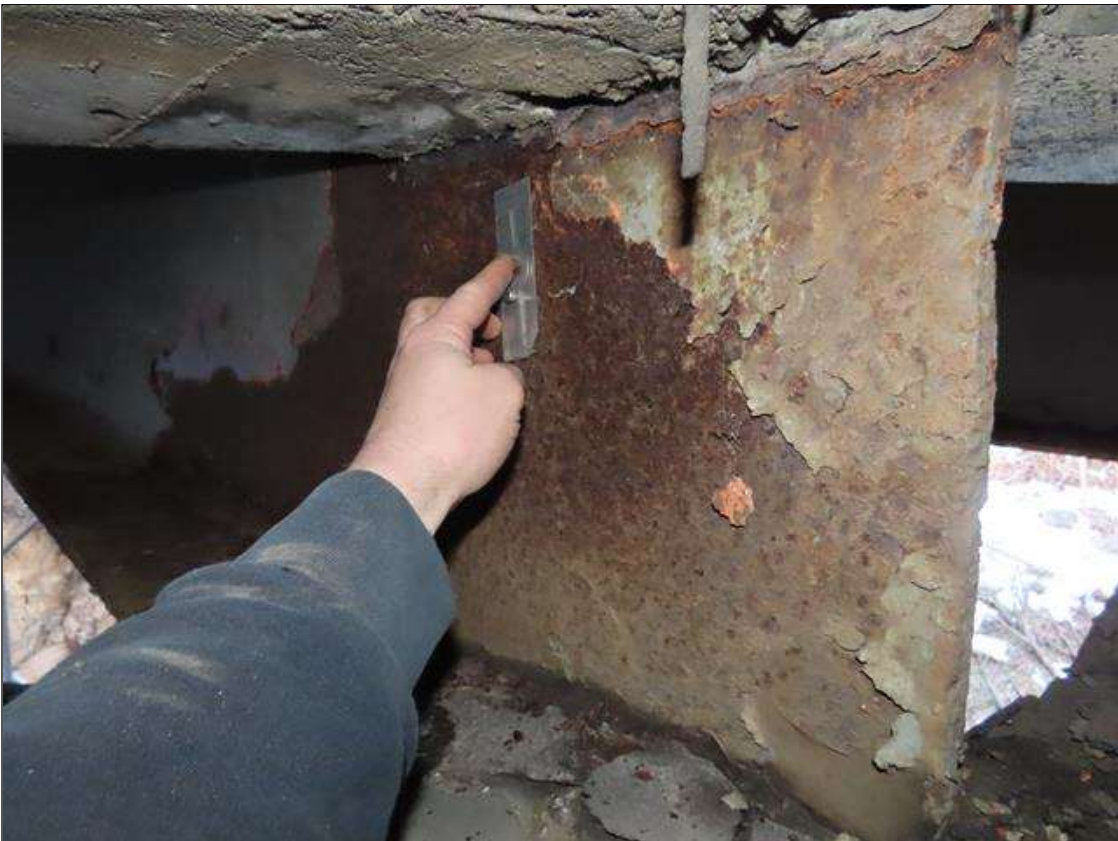
SPAN 3 BEAM 10 - WEB SECTION LOSS (UP TO 1/8IN SL, 1/2IN REMAIN) TO FULL HEIGHT X 24IN L. AT NEAR END DIAPHRAGM
