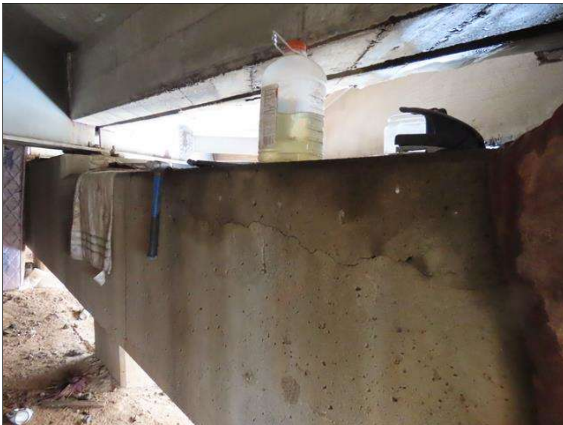
BENT 1 CAP - DELAMINATION (9FT L. X 10IN H.) TO NEAR FACE AT TOP CORNER BELOW BAY 10
