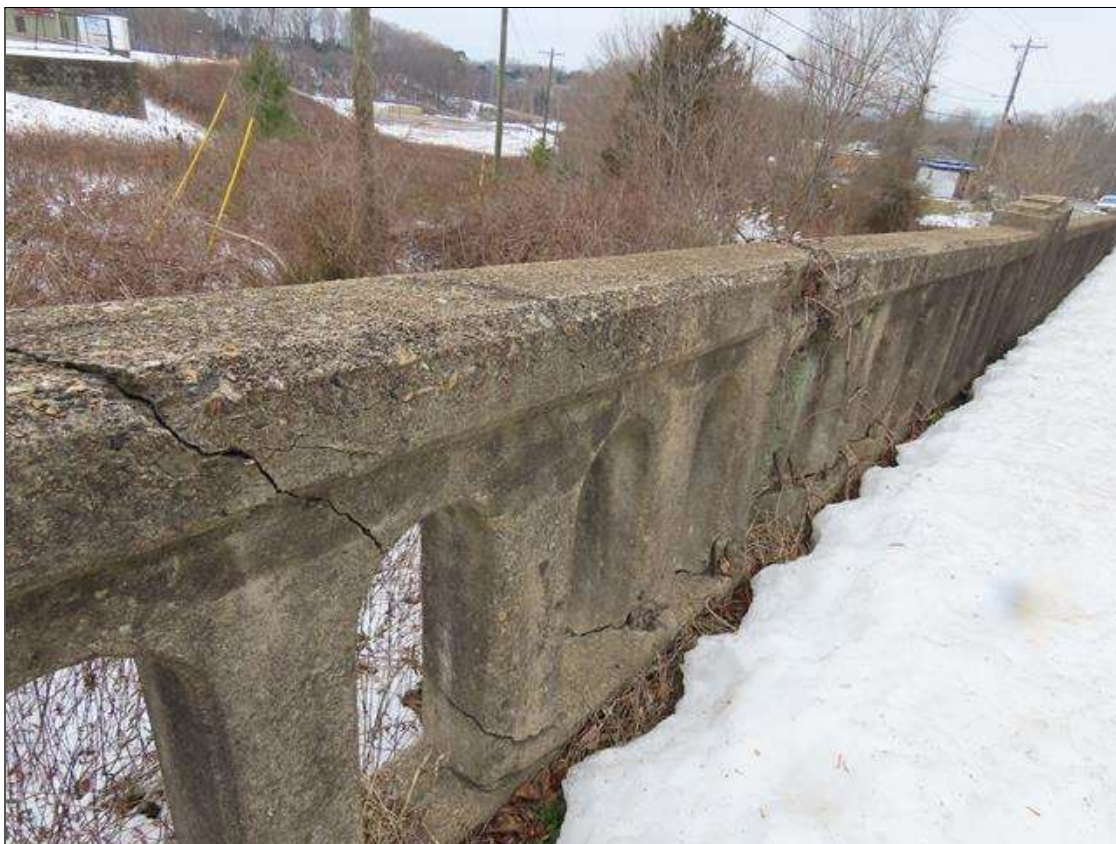
SPAN 5 RIGHT RAIL - HEAVY IMPACT DAMAGE (FULL HEIGHT X 10FT L.) WITH BROKEN/SPALLED CONCRETE & EXPOSED REBAR STARTING 5FT FROM NEAR END (PAR PHOTO 1/2)
