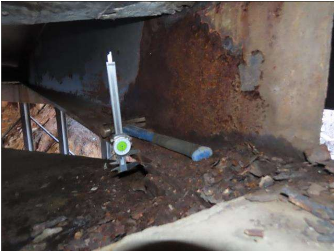
SPAN 3 BEAM 9 - BOTTOM FLANGE SECTION LOSS (UP TO 20% SL, 3/16IN SL, 3/4IN REMAIN) TO FULL WIDTH FOR 3FT AT NEAR END
