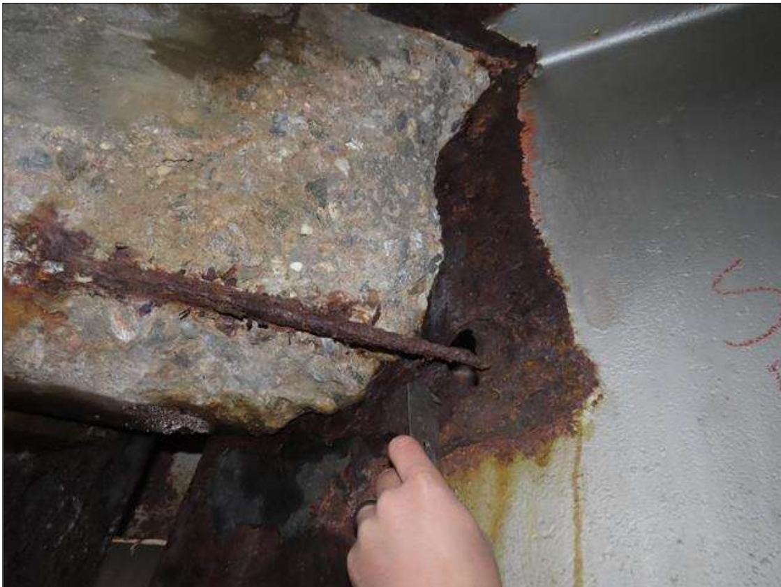
SPAN 5 BEAM 7 - WEB SECTION LOSS (UP TO 100%, AVG. 1/8IN REMAIN) FOR 18IN L. X 25IN H. AT NEAR END DIAPHRAGM (PAR PHOTO)
