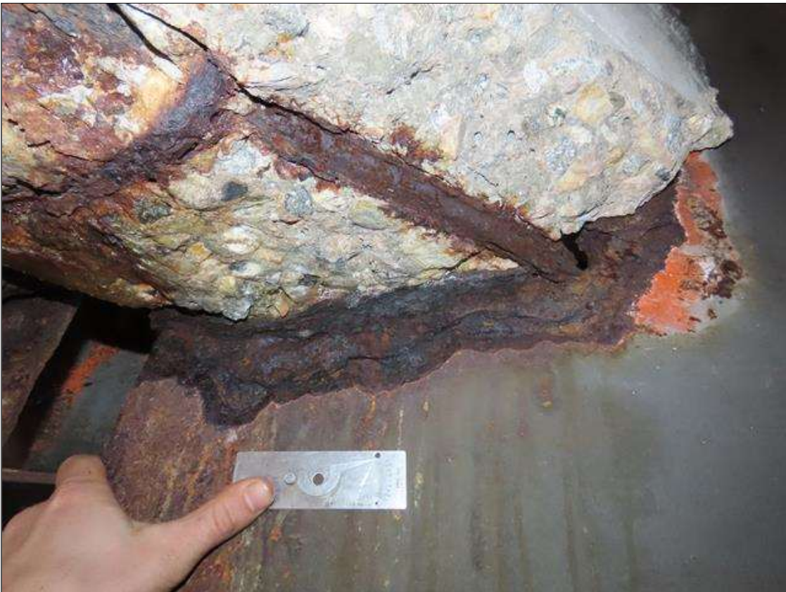
SPAN 4 BEAM 7 - WEB SECTION LOSS (7/16IN SL, 1/8IN REMAIN) FOR 16IN L. X 6IN H. AT NEAR END DIAPHRAGM (PAR PHOTO)
