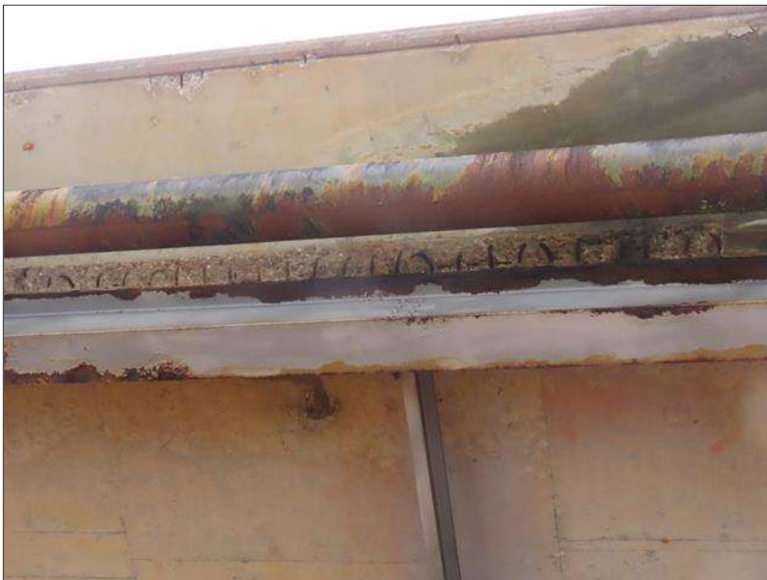
SPAN 2 DECK - SPALL (15FT X 8IN X 3IN) WITH EXPOSED REBAR TO RIGHT SIDE OF BEAM 11 HAUNCH AT MIDSPAN (PAR PHOTO)
