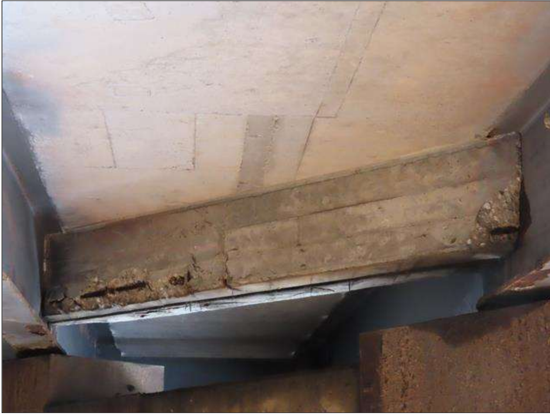
SPAN 2 BAY 9 FAR DIAPHRAGM - 2X SPALLS (UP TO 48IN X 12IN X 3IN) WITH EXPOSED REBAR THROUGHOUT (PAR PHOTO)
