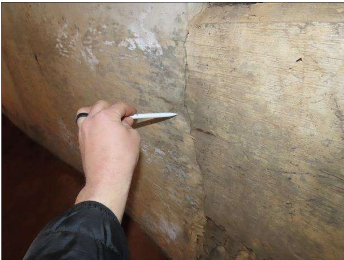
END BENT 2 CAP - VERTICAL CRACK (1/16IN X FULL HEIGHT) TO FACE BELOW BAY 5
