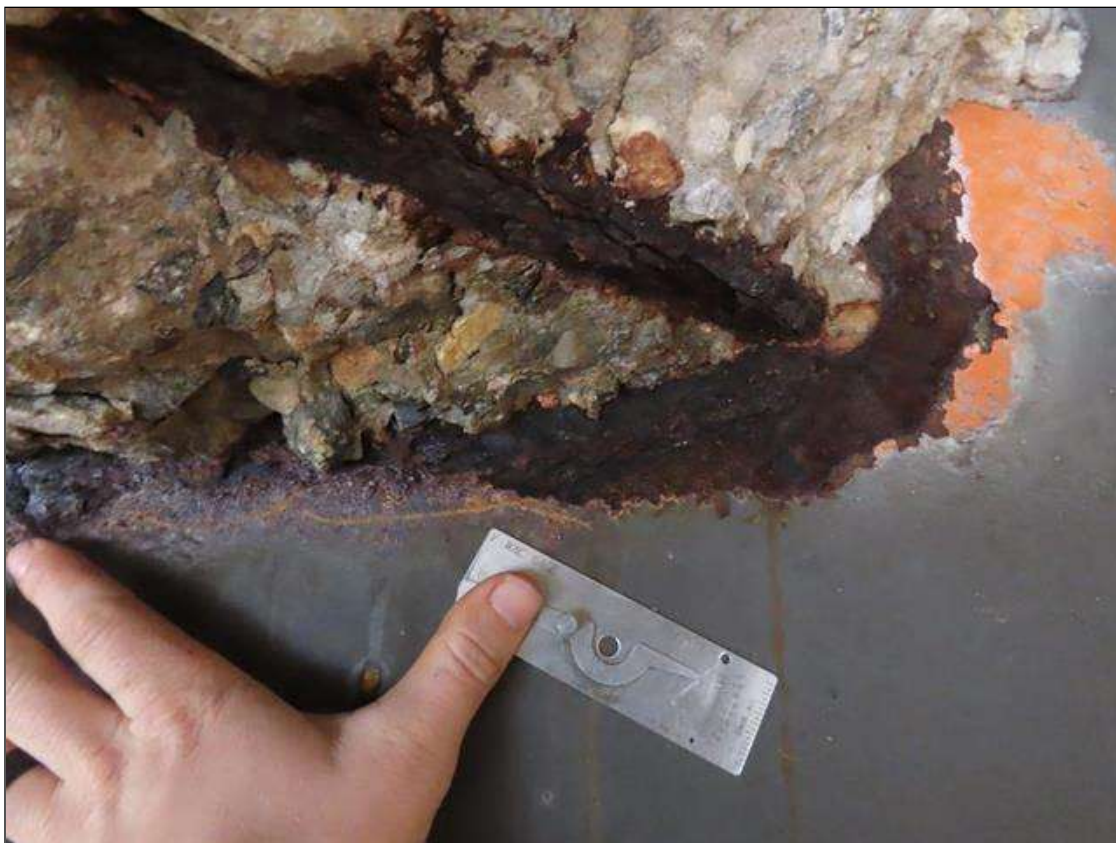
SPAN 4 BEAM 8 - WEB SECTION LOSS (1/4IN SL, 3/8IN REMAIN) FOR 12IN L. X 3IN H. AT NEAR END DIAPHRAGM (PAR PHOTO)
