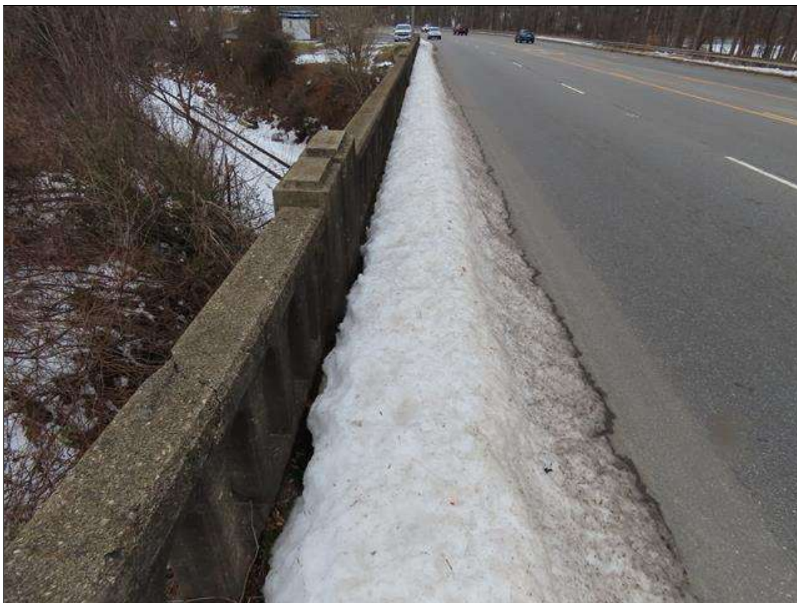
SPAN 5 DECK - SNOW/ICE PACKED THROUGHOUT RIGHT SIDE RAIL CURB
