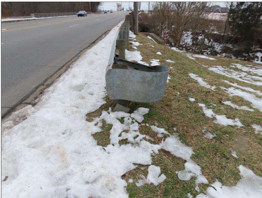
NEAR RIGHT GUARDRAIL END TREATMENT - MODERATE IMPACT DAMAGE
