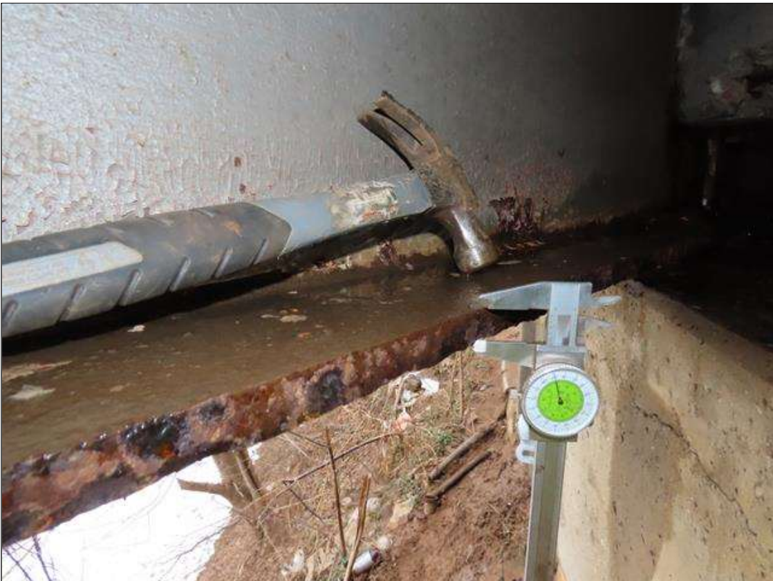
SPAN 2 BEAM 11 - BOTTOM FLANGE SECTION LOSS (UP TO 4% SL, 1/16IN SL, 11/16IN REMAIN) TO LEFT SIDE, 5IN W. FOR 2/3 LENGTH
