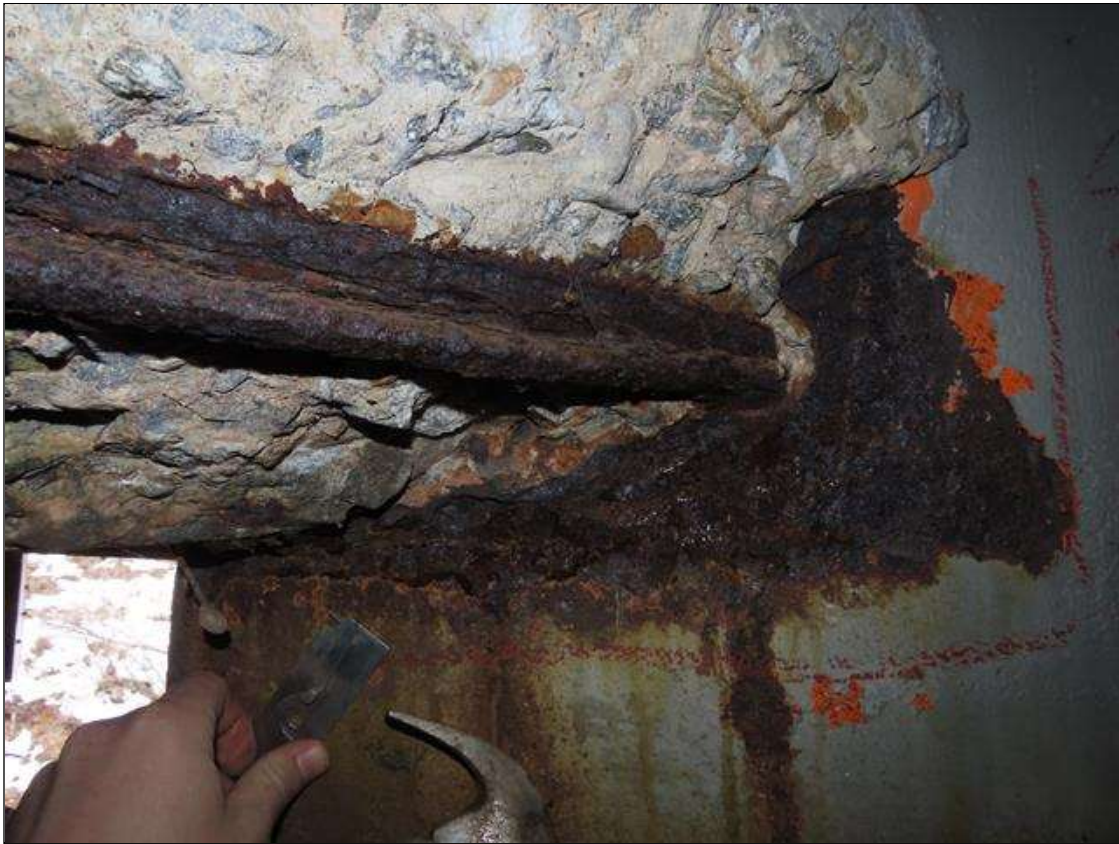
SPAN 1 BEAM 9 - WEB SECTION LOSS (UP TO 100% SL, AVG. 1/8IN REMAIN) FOR 16IN L. X 4IN H. TO FAR END DIAPHRAGM (PAR PHOTO)
