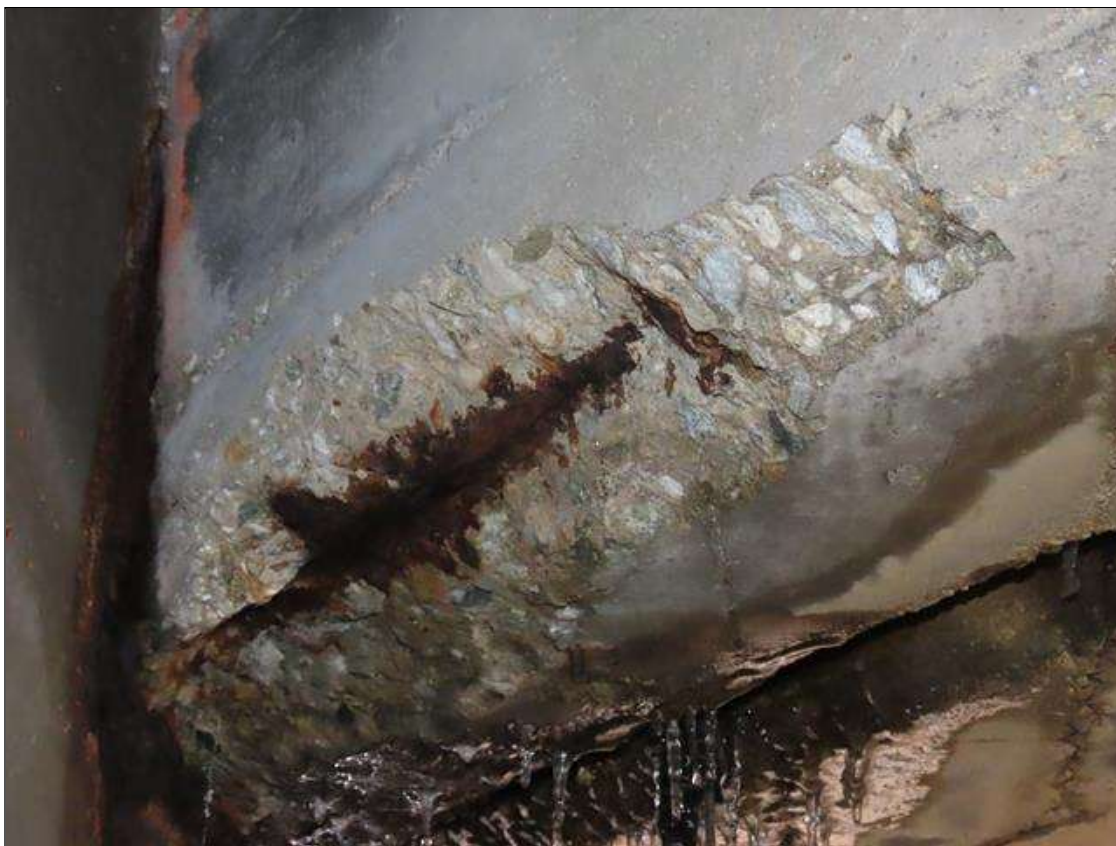
SPAN 5 BAY 10 NEAR DIAPHRAGM - SPALL (24IN X 8IN X 3IN) WITH EXPOSED REBAR ADJACENT TO BEAM 11 (PAR PHOTO)
