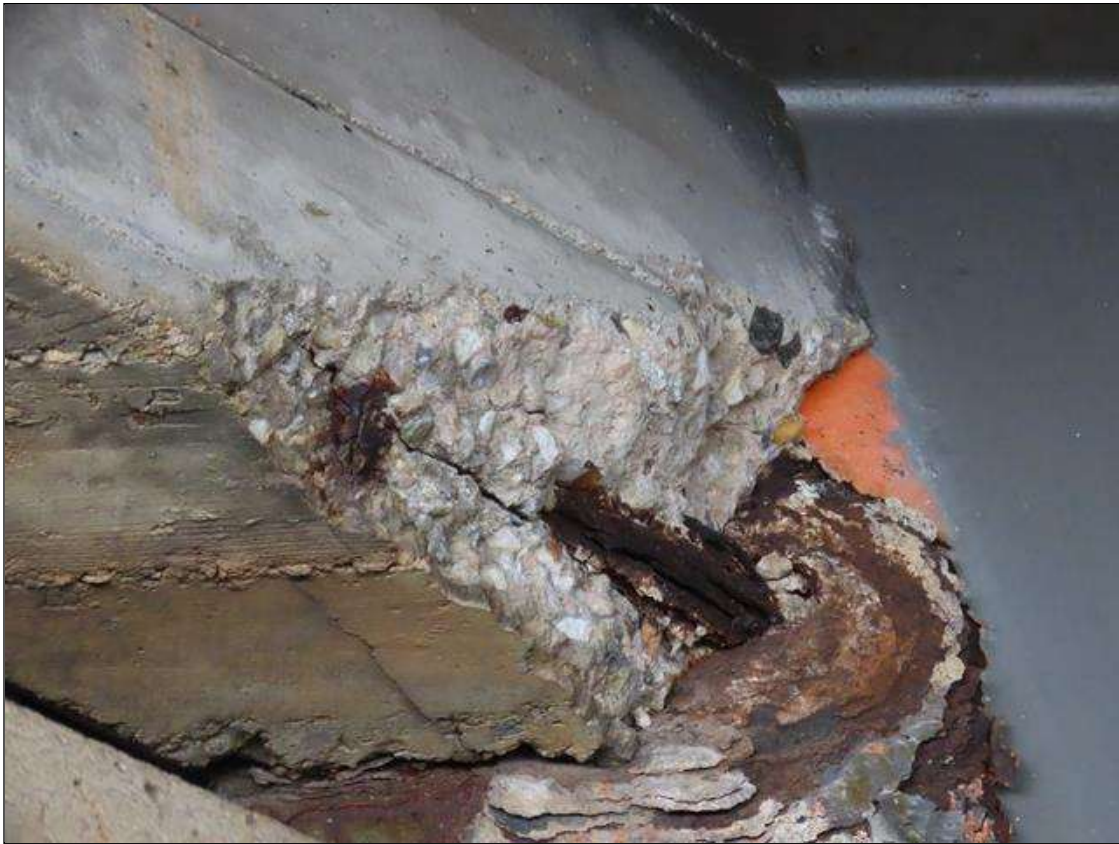
SPAN 4 BAY 8 FAR DIAPHRAGM - SPALL (16IN X 10IN X 4IN) WITH EXPOSED REBAR ADJACENT TO BEAM 9 (PAR PHOTO)
