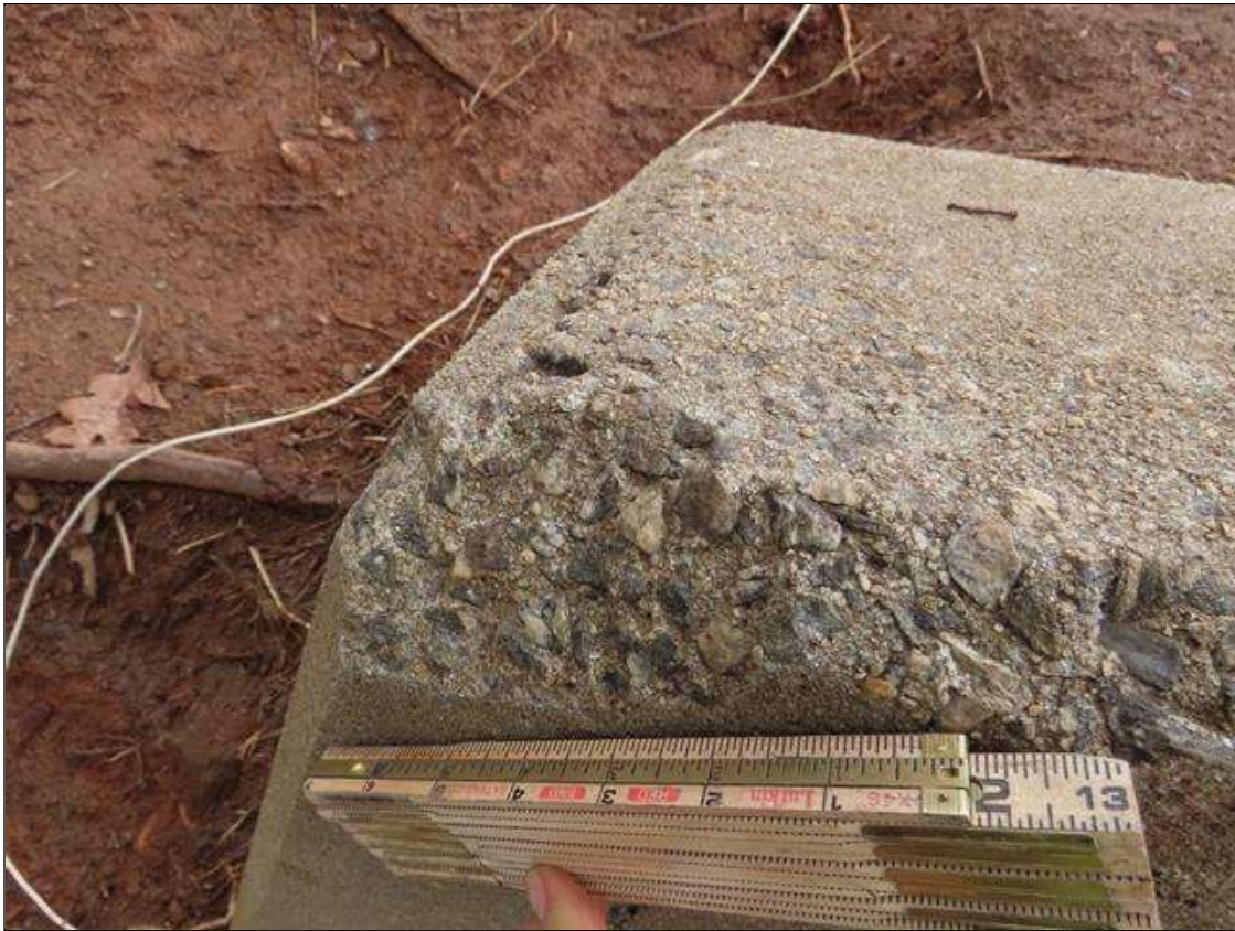
FAR LEFT WINGWALL - SPALL (6IN X 4IN X 1IN) WITH NO EXPOSED REBAR TO TOP CORNER AT LEFT SIDE (FAR RIGHT WINGWALL SIMILAR, AT RIGHT SIDE TOP)
