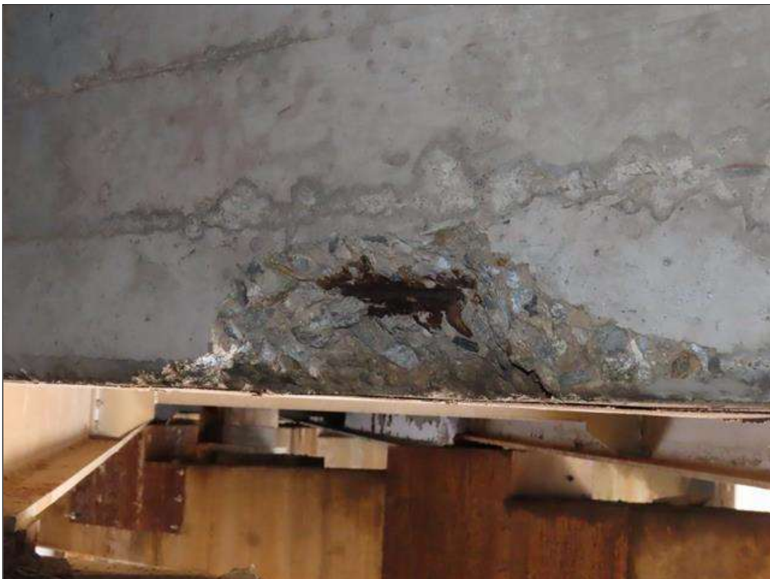
SPAN 1 BAY 8 FAR DIAPHRAGM - SPALL (24IN X 8IN X 4IN) WITH EXPOSED REBAR AT MIDDLE (PAR PHOTO)
