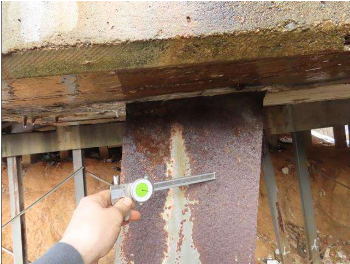
BENT 3 PILE 17 - FAR FLANGE SECTION LOSS (1/8IN SL, 5/16IN REMAIN) TO FULL WIDTH X 4IN H. AT TOP (NEAR FLANGE SIMILAR) (PAR PHOTO)
