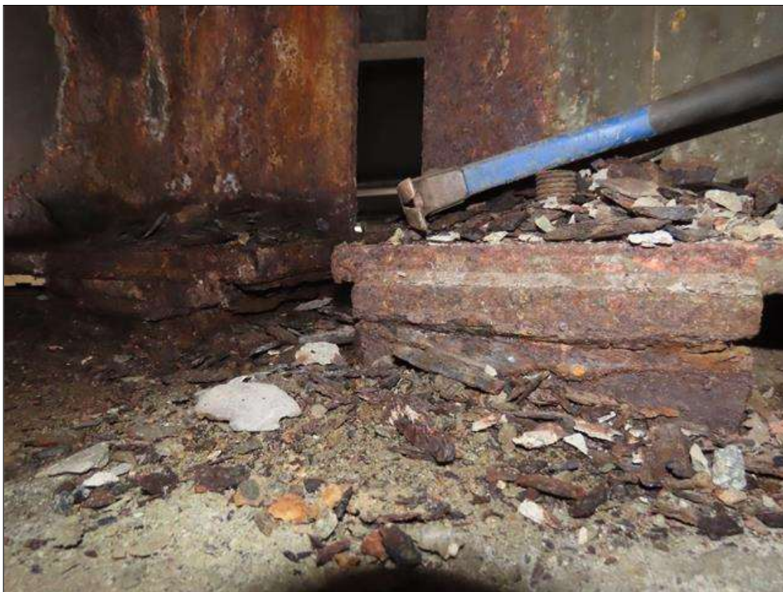
TYP. HEAVY SCALING TO BEARINGS AT BENT 3, BEAMLIN 7
