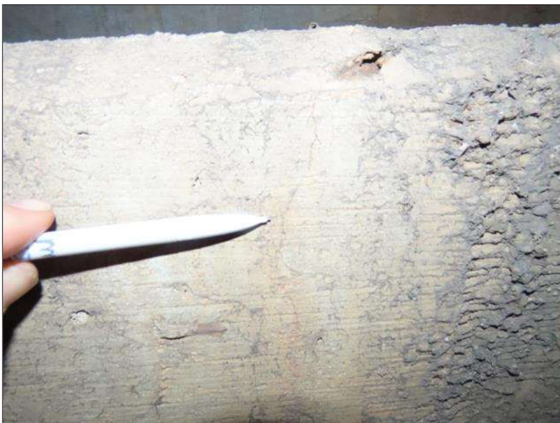
TYP. INTERMITTENT VERTICAL HAIRLINE CRACKING (UP TO FULL HEIGHT) THROUGHOUT END BENT 2 CAP, BAY 4
