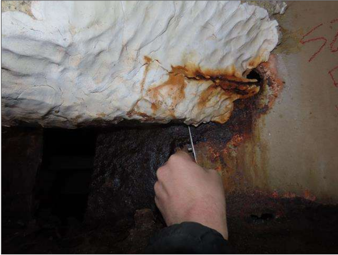
SPAN 2 BEAM 7- WEB SECTION LOSS (UP TO 100%, AVG. 3/16IN REMAIN) FOR 16IN L. X 8IN H. AT NEAR END DIAPHRAGM (PAR PHOTO)
