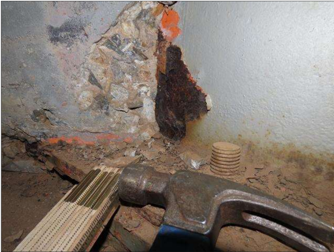
SPAN 1 BEAM 7 - WEB SECTION LOSS (1/16IN SL, 7/16IN REMAIN) TO RIGHT SIDE, 3IN X 3IN AT NEAR END BOTTOM
