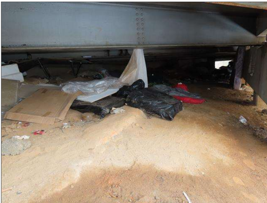
HEAVY DEBRIS & VAGRANT QUARTERS THROUGHOUT SPAN 1 OF BRIDGE, UNABLE TO OBTAIN FULL END BENT 1 PHOTO (PHOTO 2/2)
