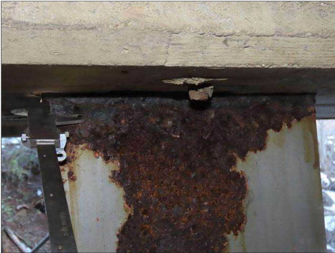
BENT 2 PILE 10 - NEAR FLANGE SECTION LOSS (UP TO 100% SL, AVG. 1/4IN REMAIN) TO FULL WIDTH X 3IN H. AT TOP (FAR FLANGE SIMILAR) (PAR PHOTO)
