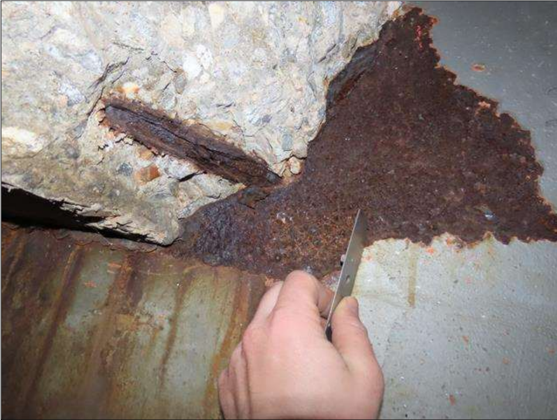
SPAN 2 BEAM 10 - WEB SECTION LOSS (UP TO 3/8IN SL, 1/8IN REMAIN) FOR 18IN L. X 10IN H. AT FAR END DIAPHRAGM (PAR PHOTO)
