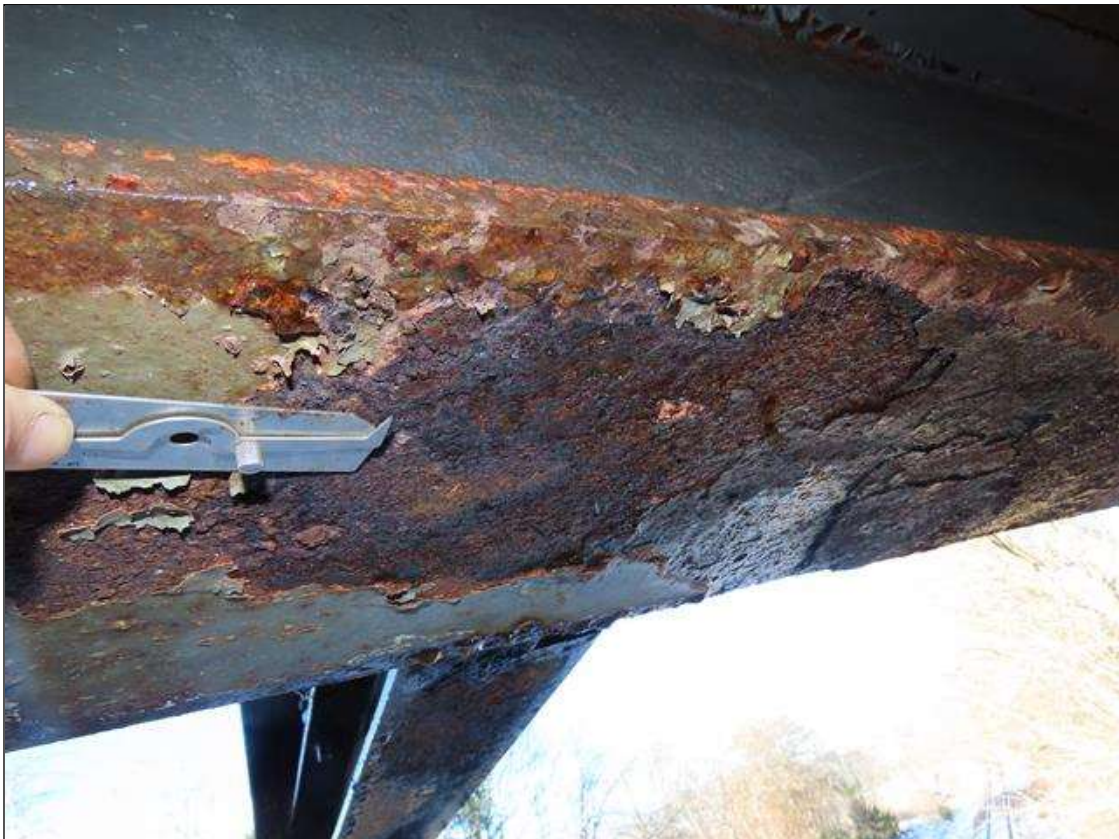
SPAN 2 BEAM 11 - BOTTOM FLANGE SECTION LOSS (UP TO 8% SL, 1/16IN SL, 11/16IN REMAIN) TO FULL WIDTH FOR 4FT L. AT FAR END
