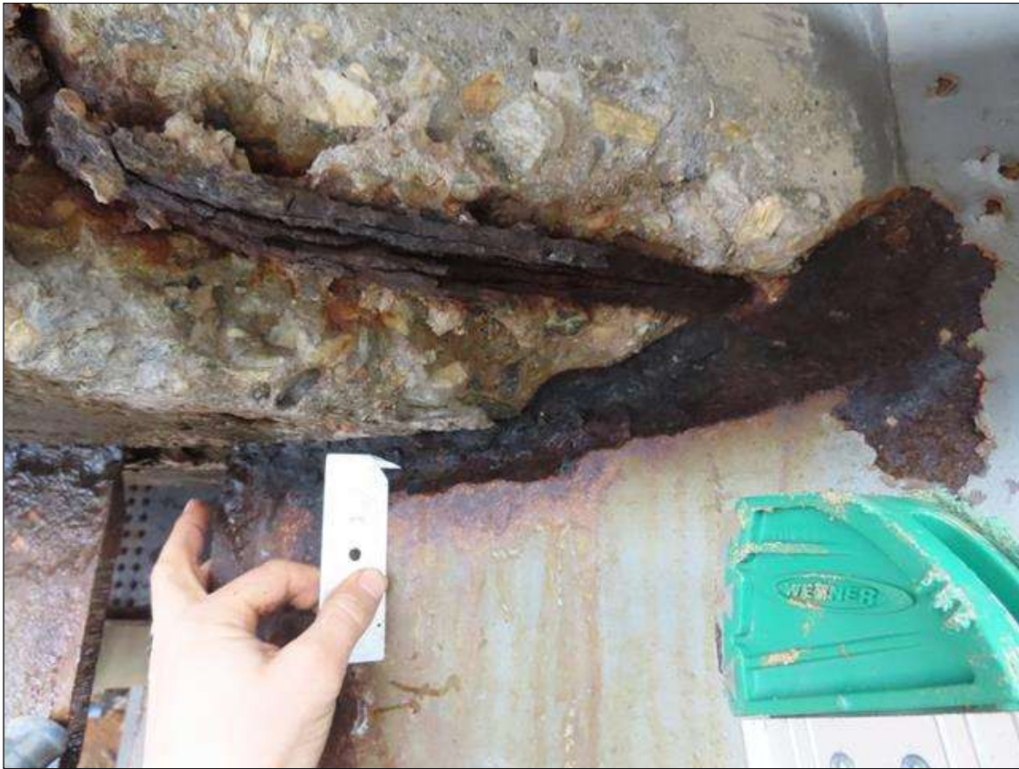
SPAN 4 BEAM 11 - WEB SECTION LOSS (7/16IN SL, 1/8IN REMAIN) FOR 18IN L. X 3IN H. AT NEAR END DIAPHRAGM (PAR PHOTO)
