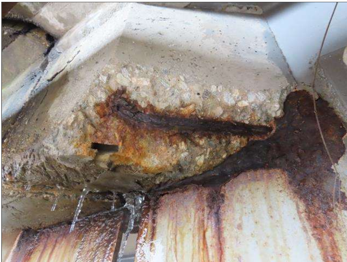
SPAN 5 RIGHT OVERHANG DIAPHRAGM AT NEAR END - SPALL (14IN X 8IN X 2IN) WITH EXPOSED REBAR (PAR PHOTO)
