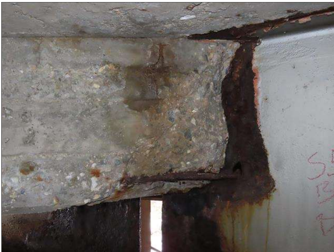
SPAN 5 BAY 7 NEAR DIAPHRAGM - SPALL (20IN X 20IN X 4IN) WITH EXPOSED REBAR ADJACENT TO BEAM 7 (PAR PHOTO)
