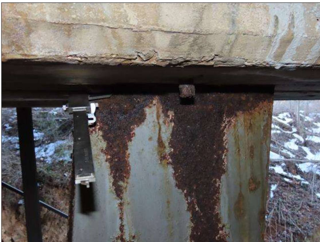
BENT 2 PILE 9 - NEAR FLANGE SECTION LOSS (3/16IN SL, 1/4IN REMAIN) AT TOP, 2IN H. X FULL WIDTH (SIMILAR AT FAR FLANGE) (PAR PHOTO)
