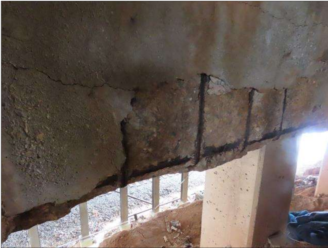
BENT 4 CAP - DELAMINATION (FULL HEIGHT) & 2X SPALLS (UP TO 48IN X 16IN X 3IN) WITH EXPOSED REBAR TO FAR FACE BELOW BAYS 8-10 (25FT TOTAL) (PAR PHOTO 3/3)
