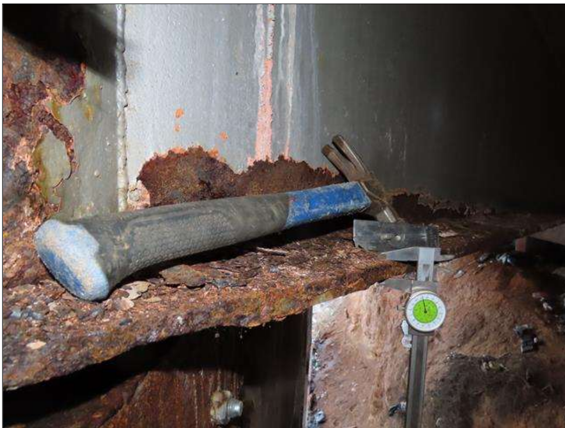
SPAN 2 BEAM 7 - BOTTOM FLANGE SECTION LOSS (UP TO 25% SL, 3/16IN SL, 9/16IN REMAIN) TO FULL WIDTH FOR 4FT L. & WEB SECTION LOSS (1/8IN SL, 3/8IN REMAIN) TO BOTTOM X 2IN H. FOR 4FT AT FAR END (PAR PHOTO)
