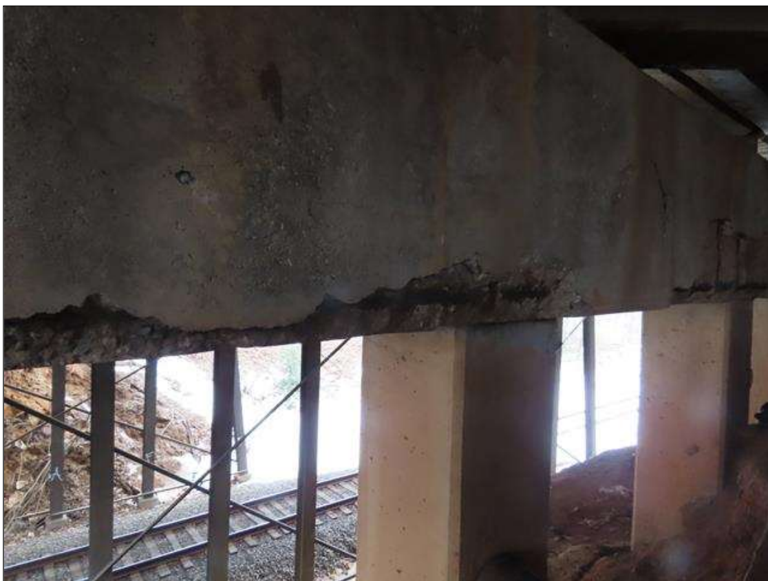
BENT 4 CAP - DELAMINATION (FULL HEIGHT) & 2X SPALLS (UP TO 48IN X 16IN X 3IN) WITH EXPOSED REBAR TO FAR FACE BELOW BAYS 8-10 (25FT TOTAL) (PAR PHOTO 2/3)
