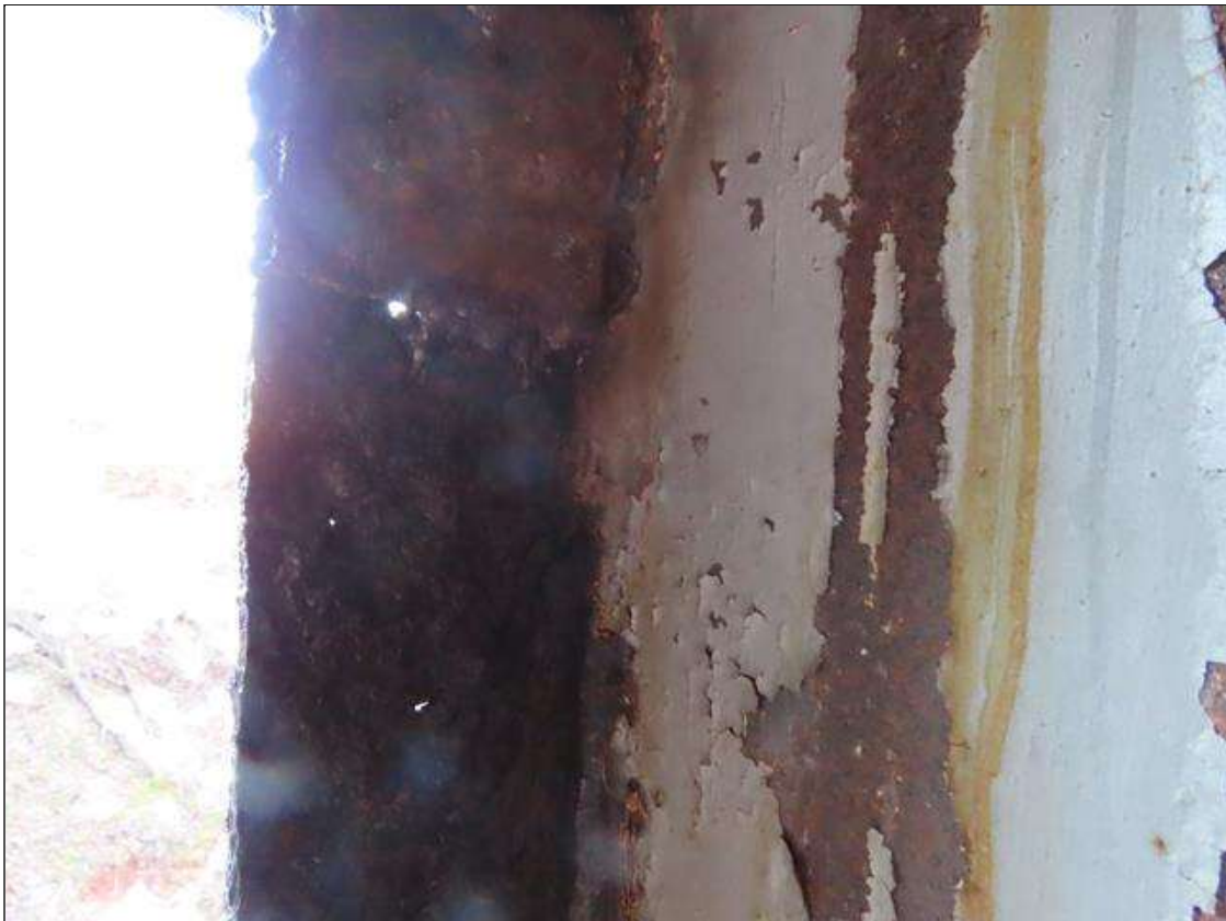
BENT 2 PILE 15 - NEAR & FAR FLANGE SECTION LOSS (UP TO 100% SL, AVG. 1/4IN REMAIN) TO FULL WIDTH, 4IN H. AT NEAR FLANGE, 4FT H. AT FAR FLANGE UNDER REAIR (PAR PHOTO 2/2)
