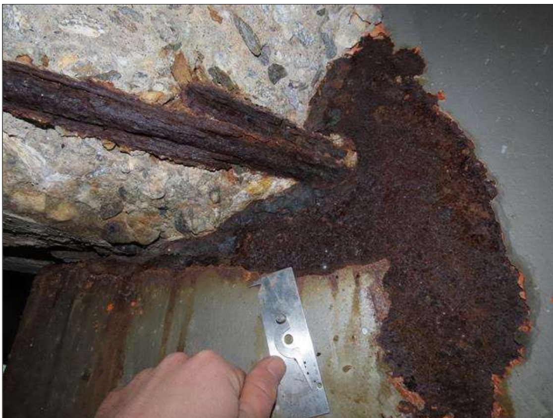
SPAN 2 BEAM 9 - WEB SECTION LOSS (UP TO 100% SL, AVG. 1/8IN REMAIN) FOR 15IN L. X 8IN H. AT FAR END DIAPHRAGM (PAR PHOTO)
