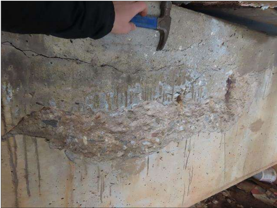
BENT 1 CAP - SPALL (36IN X 12IN X 2IN) WITH EXPOSED REBAR TO FAR FACE BELOW BEAM 9 (PAR PHOTO)
