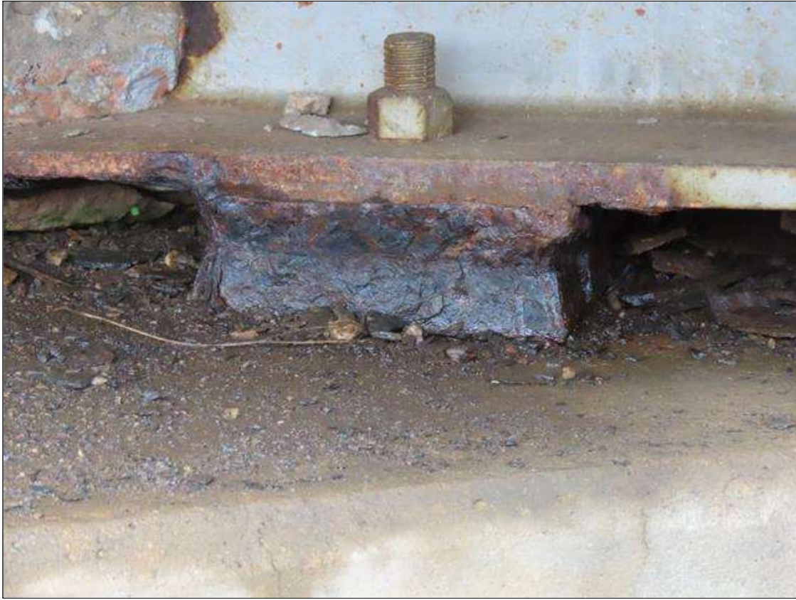
SPAN 1 BEAM 11 NEAR BEARING - HEAVY SCALING THROUGHOUT
