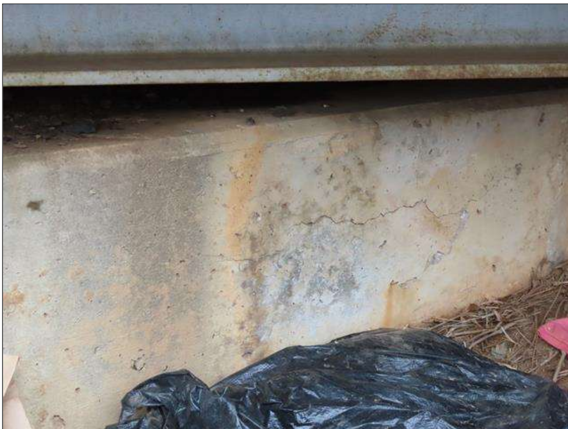
END BENT 1 CAP - DELAMINATION (24IN X 10IN) TO FACE BELOW BEAM 11
