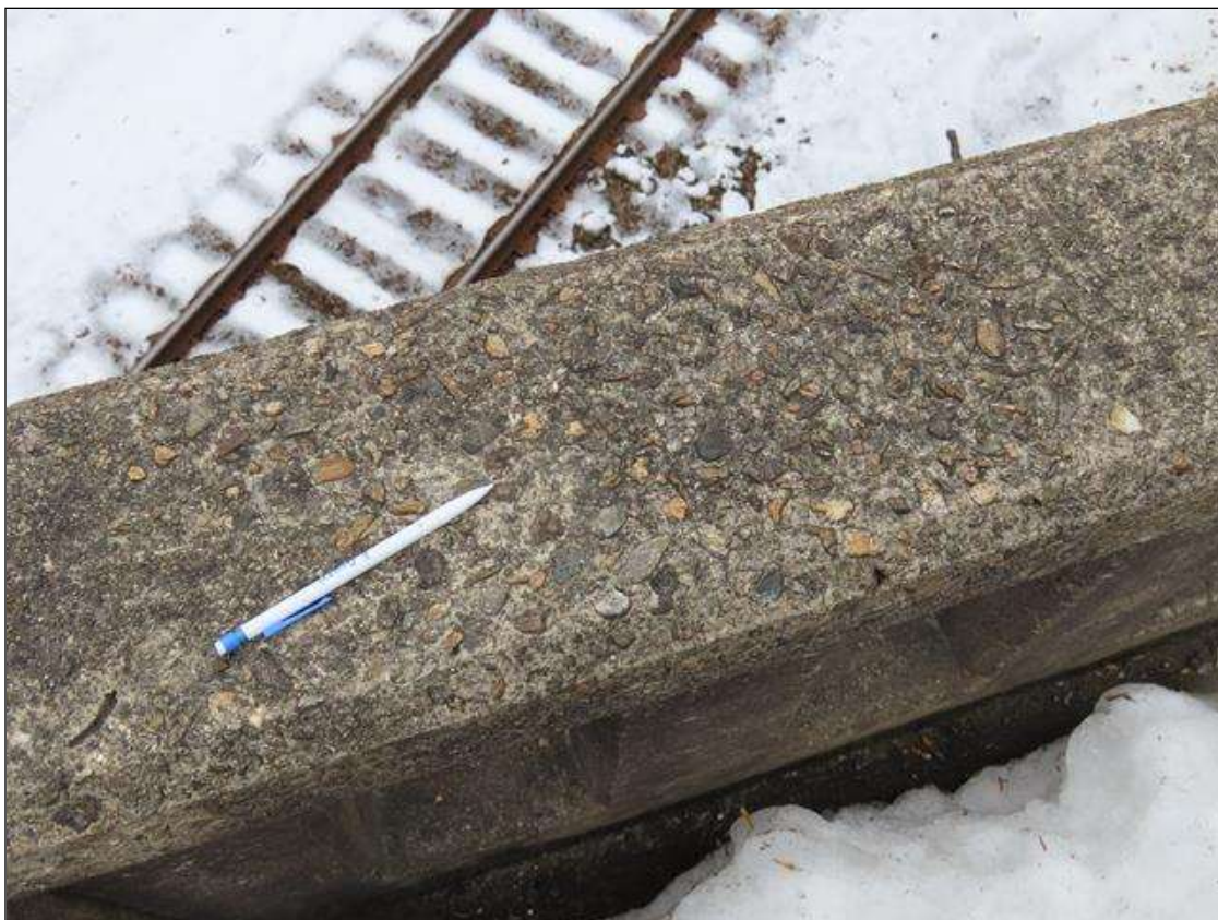
TYP. MINOR WEATHERING WITH EXPOSED COARSE AGGREGATE THROUGHOUT RAILS, SPAN 2 RIGHT RAIL
