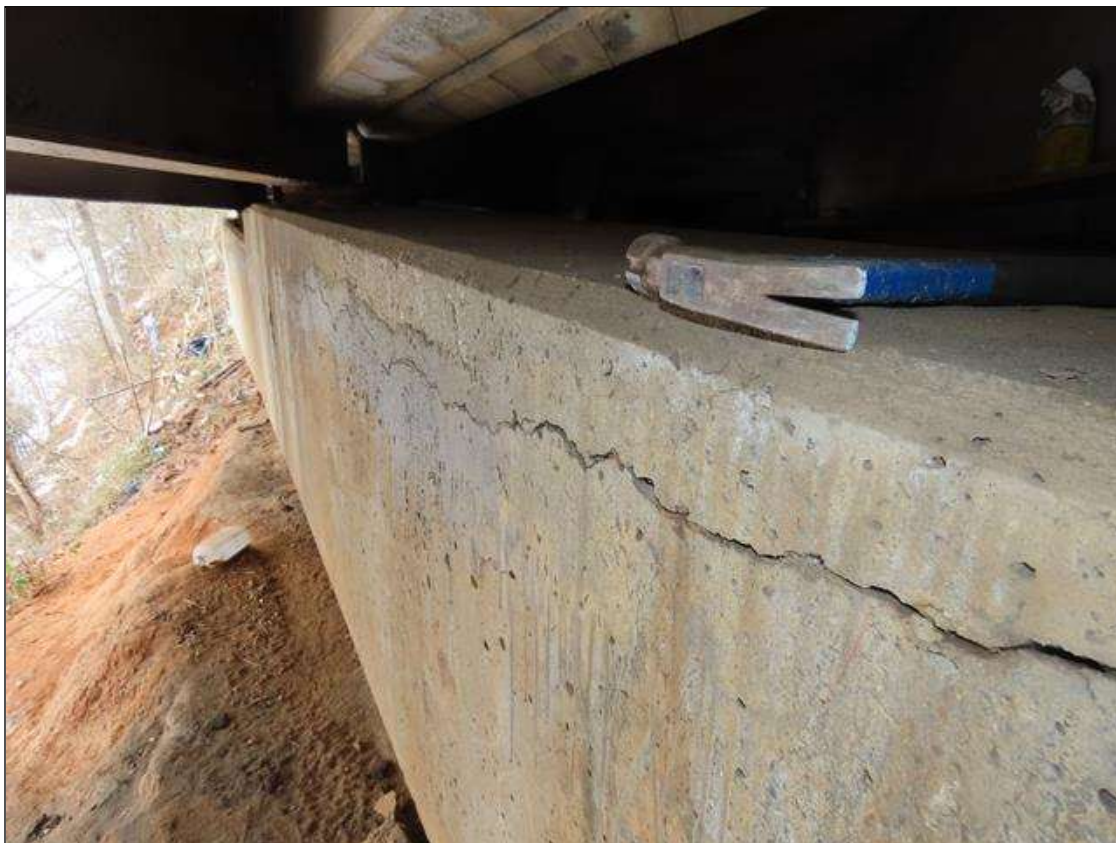
BENT 1 CAP - DELAMINATION (35FT L. X UP TO 24IN H.) TO FAR FACE AT TOP BELOW BAYS 7-11 (PAR PHOTO)
