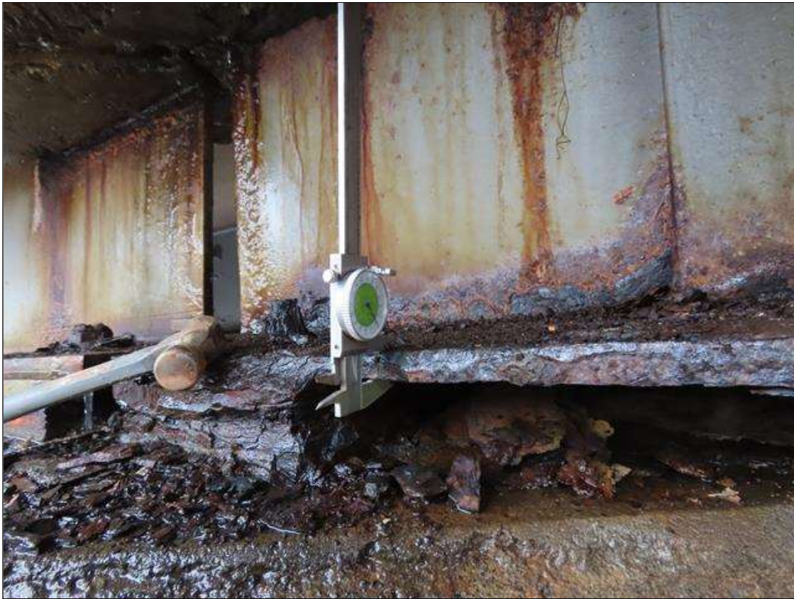
SPAN 5 BEAM 11 - BOTTOM FLANGE SECTION LOSS (UP TO 29% SL, 1/4IN SL, 5/8IN REMAIN) TO FULL WIDTH FOR 2FT L. & WEB SECTION LOSS (1/8IN SL, 7/16IN REMAIN) TO BOTTOM X 2IN H. FOR 2FT L. AT NEAR END (PAR PHOTO)
