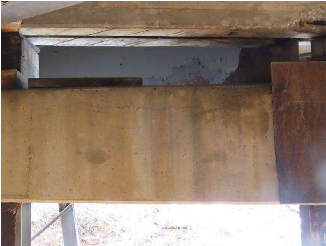
BENT 2 CAP - HORIZONTAL CRACK (1/32IN X 4.5FT L.) TO NEAR FACE AT TOP BELOW BAY 8
