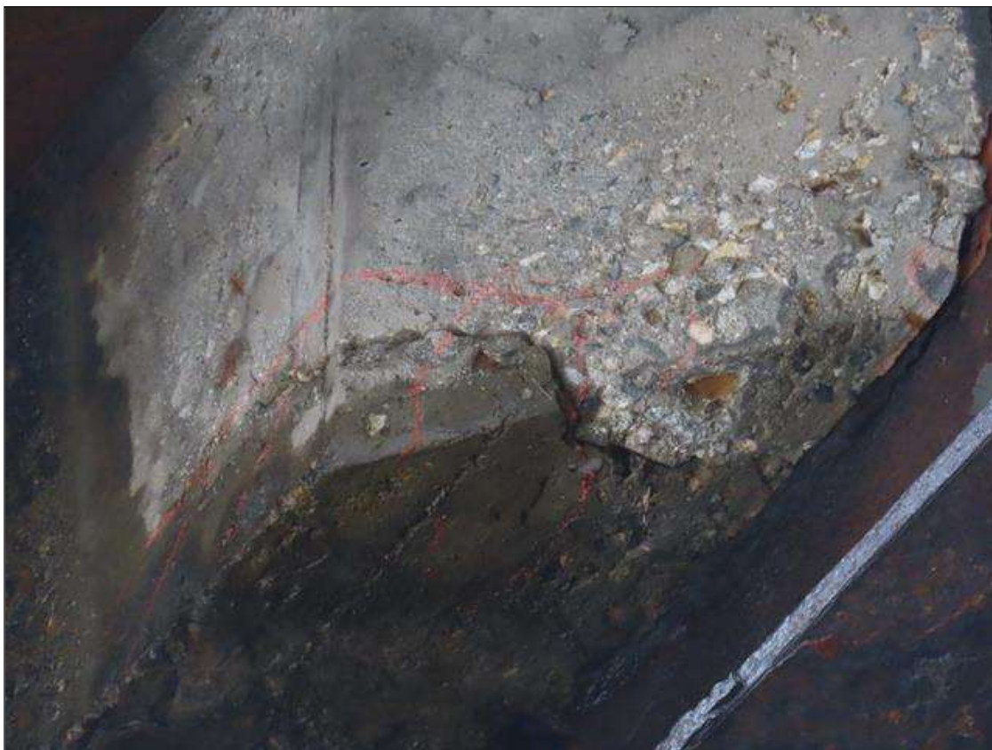
SPAN 3 RIGHT OVERHANG DIAPHRAGM AT NEAR END - DELAMINATION (1SQ. FT.) THROUGHOUT
