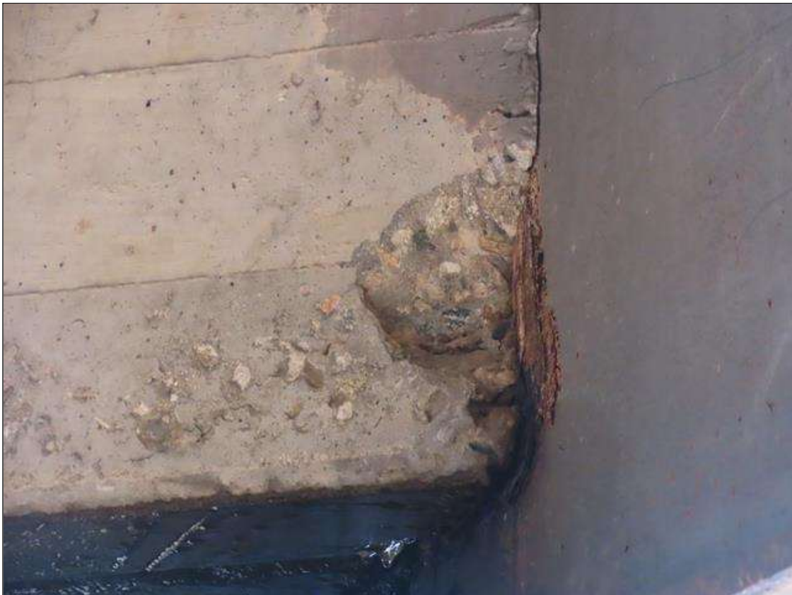
SPAN 2 BAY 10 FAR DIAPHRAGM - SPALL (6IN DIA. X 2IN D.) WITH NO EXPOSED REBAR ADJACENT TO BEAM
