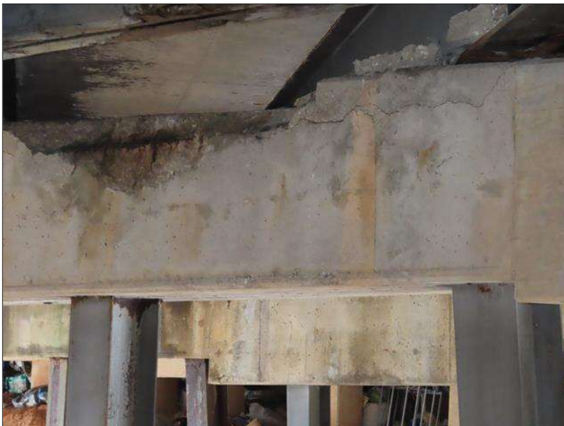
BENT 3 CAP - SPALL & DELAMINATION (9FT L. X 18IN H. X UP TO 6IN D.) WITH EXPOSED REBAR TO FAR FACE & TOP BELOW BAY 7 (PAR PHOTO)
