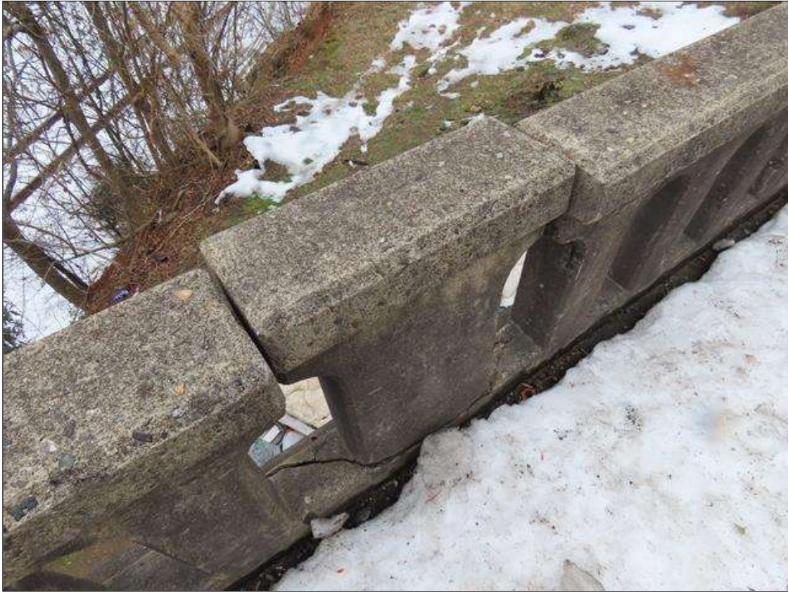
SPAN 1 RIGHT RAIL - HEAVY IMPACT DAMAGE (2FTL. X FULL HEIGHT) WITH BROKEN CONCRETE AND LEANING RAIL AT MIDSPAN (PAR PHOTO)
