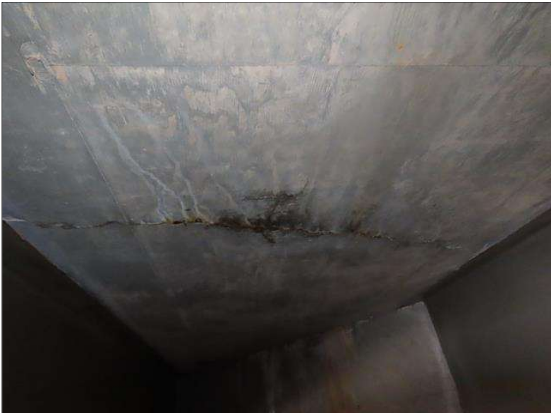
SPAN 5 DECK - TRANSVERSE HAIRLINE CRACK (8FT L.) WITH MODERATE EFFLORESCENCE IN BAY 5 AT MIDSPAN (SIMILAR BAY 6)
