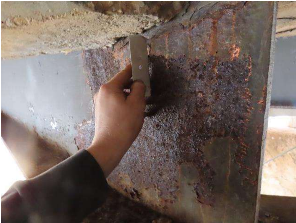
SPAN 3 BEAM 9 - WEB SECTION LOSS (3/16IN SL, 7/16IN REMAIN) FOR 18IN L. X 4IN H. AT FAR END DIAPHRAGM (PAR PHOTO)
