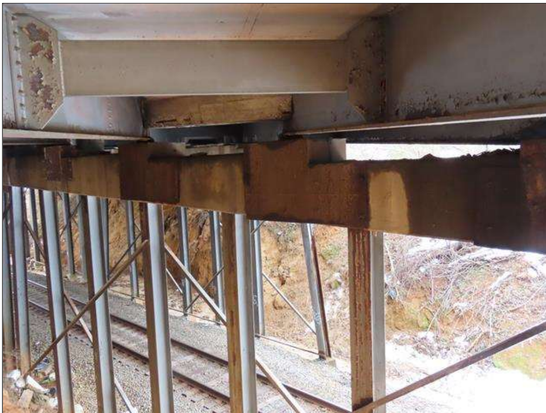
BENT 2 CAP - STEEL REPAIR PLATES (UP TO 6FT X FULL HEIGHT) (5X TOTAL) TO NEAR FACE BELOW BEAMS 7-11
