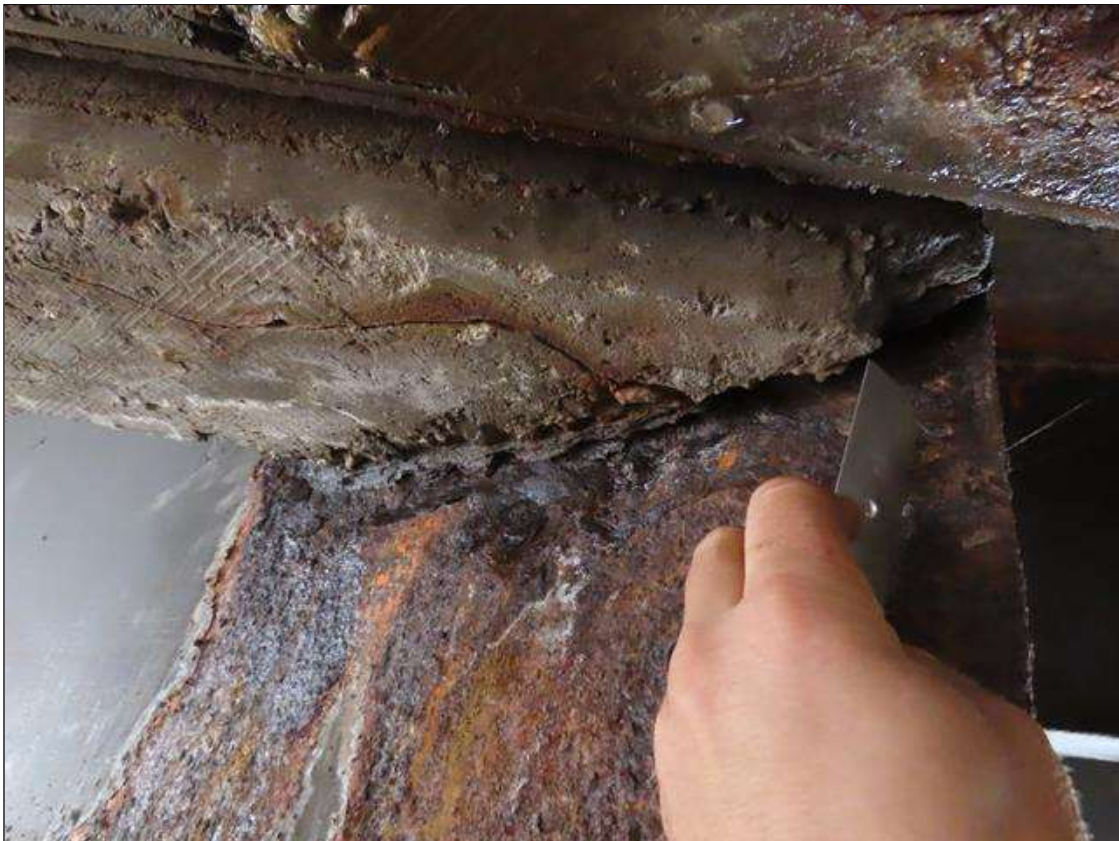
SPAN 3 BEAM 7 - WEB SECTION LOSS (UP TO 7/16IN SL, 1/8IN REMAIN) FOR 24IN L. X 5IN H. AT FAR END DIAPHRAGM (PAR PHOTO)
