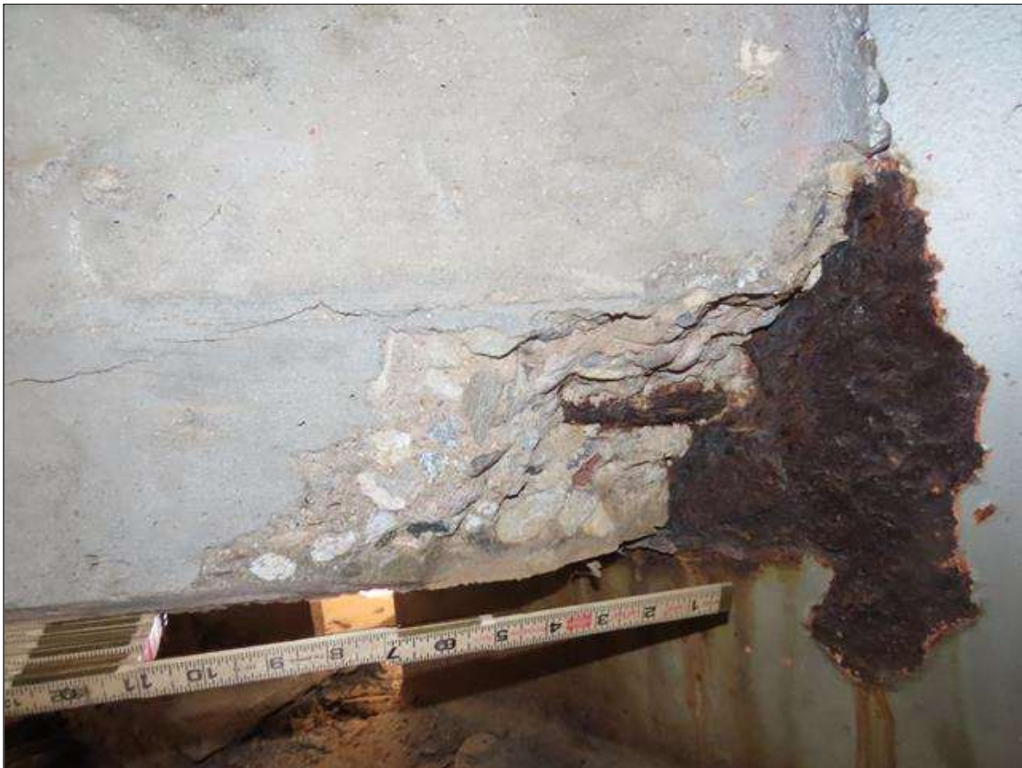
SPAN 1 BAY 9 FAR DIAPHRAGM - SPALL (12IN X 6IN 4IN) WITH EXPOSED REBAR ADJACENT TO BEAM 10 (PAR PHOTO)
