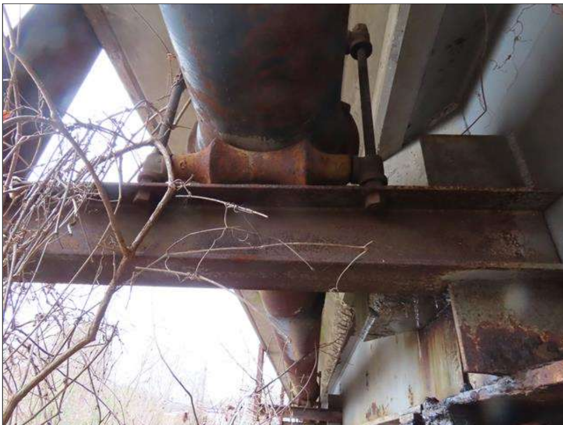
TYP. UTILITY THROUGHOUT RIGHT OVERHANG, SPAN 5 LOOKING BACK
