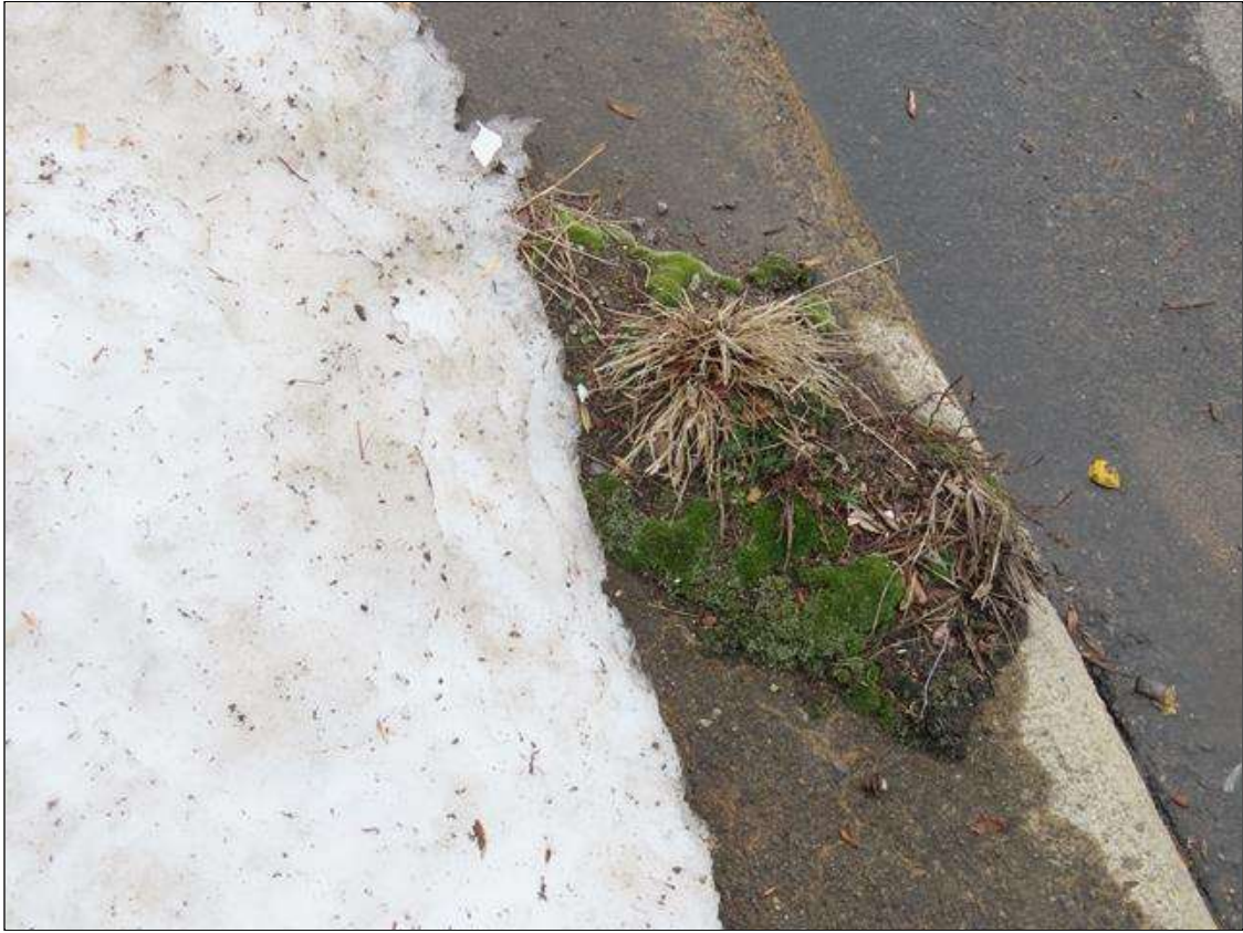
TYP. MODERATE VEGETATION GROWING AT JOINTS ON SIDEWALKS, JOINT OVER BENT 2
