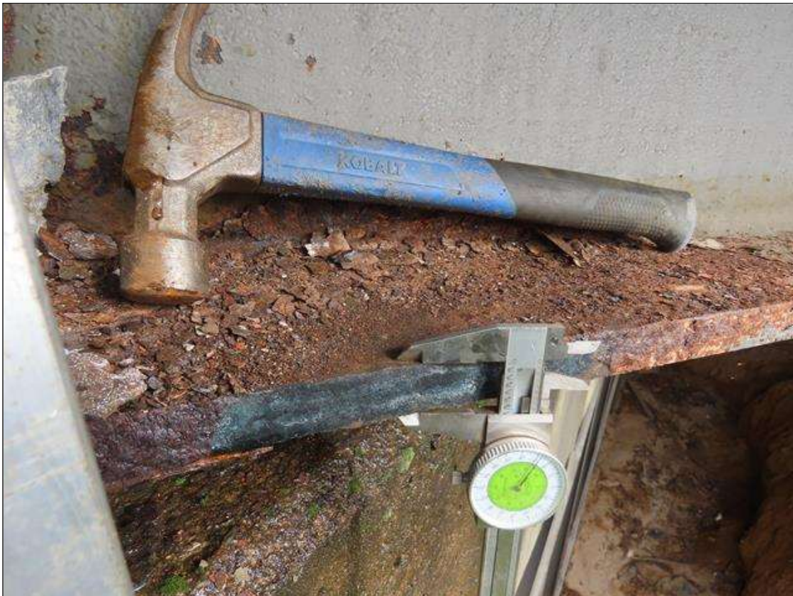
SPAN 4 BEAM 11 - BOTTOM FLANGE SECTION LOSS (UP TO 7% SL, 1/16IN SL, 13/16IN REMAIN) TO FULL WIDTH FOR 2FT L. AT NEAR END (SIMILAR AT MIDSPAN FOR 5FT L.)
