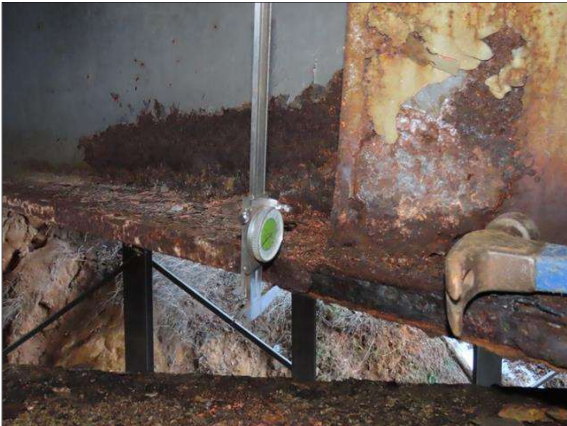
SPAN 3 BEAM 7 - BOTTOM FLANGE SECTION LOSS (UP TO 7% SL, 1/16IN SL, 13/16IN REMAIN) TO FULL WIDTH FOR 3FT AT NEAR END & WEB SCALING (NO MEASURABLE SECTION LOSS)
