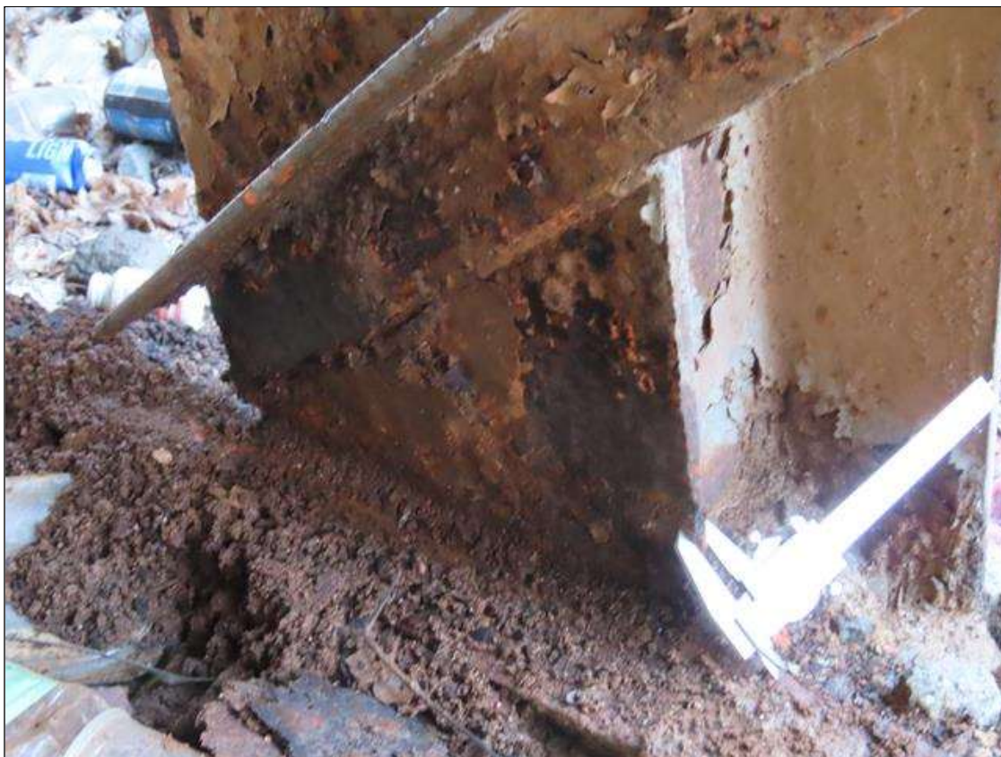
BENT 2 PILE 12 - NEAR FLANGE SECTION LOSS (1/8IN SL, 5/16IN REMAIN) TO FULL WIDTH X 1FT H. AT BOTTOM (PAR PHOTO)
