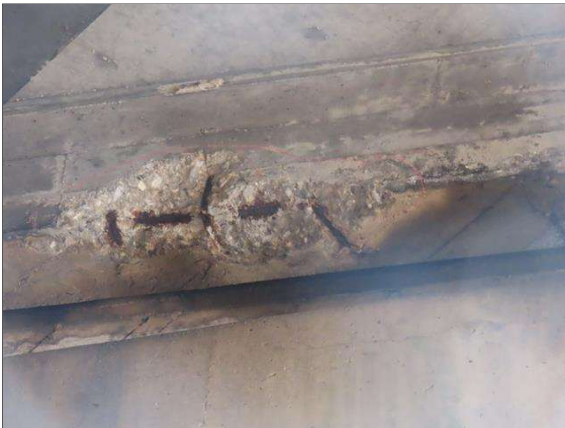
SPAN 3 BAY 10 FAR DIAPHRAGM - SPALL (36IN X 12IN X 4IN) WITH EXPOSED REBAR (PAR PHOTO)
