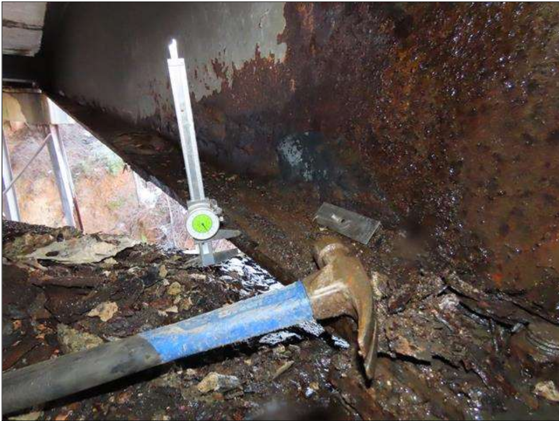
SPAN 3 BEAM 11 - BOTTOM FLANGE SECTION LOSS (UP TO 29% SL, 1/4IN SL, 5/8IN REMAIN) TO FULL WIDTH FOR 4FT L. & WEB PITTING (1/8IN PITTING, 7/16IN REMAIN) TO FULL HEIGHT (PAR PHOTO)
