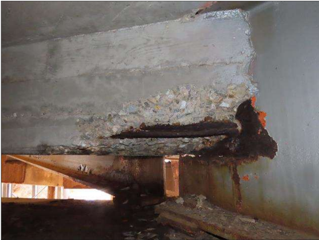
SPAN 1 BAY 8 FAR DIAPHRAGM - SPALL (30IN X 10IN X 4IN) WITH EXPOSED REBAR ADJACENT TO BEAM 9 (PAR PHOTO)
