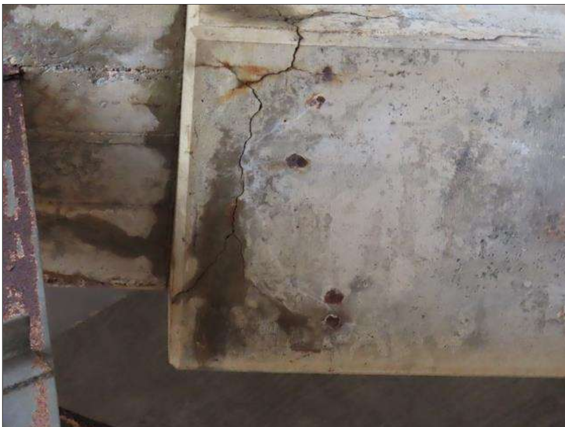
BENT 2 CAP - DELAMINATION (24IN X 8IN X 8IN) WITH MINOR RUST STAINING TO BOTTOM & FAR FACE OF CAP BETWEEN PILES 8 & 9 (PAR PHOTO)
