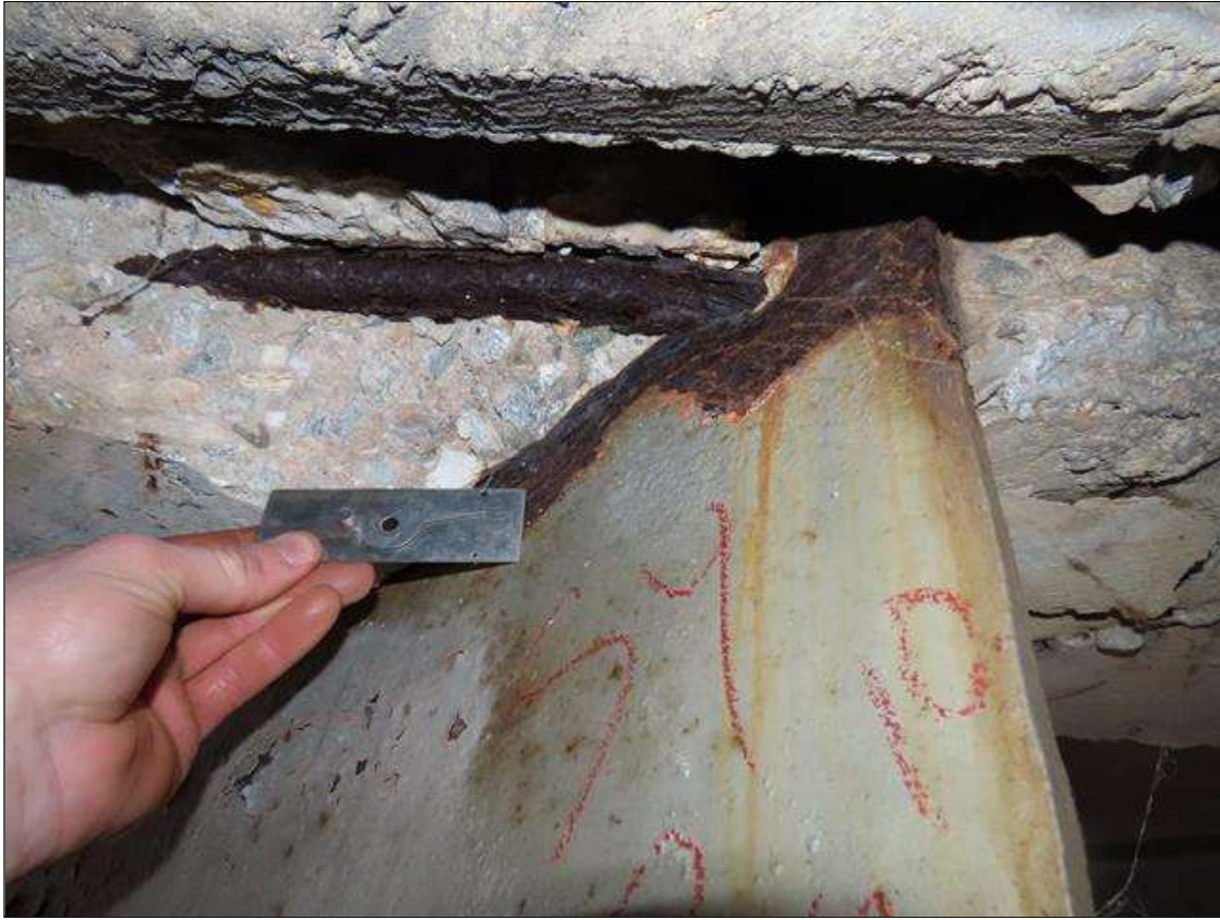
SPAN 4 BEAM 10 - WEB SECTION LOSS (1/8IN SL, 1/2IN REMAIN) FOR 8IN L. X 6IN H. AT FAR END DIAPHRAGM
