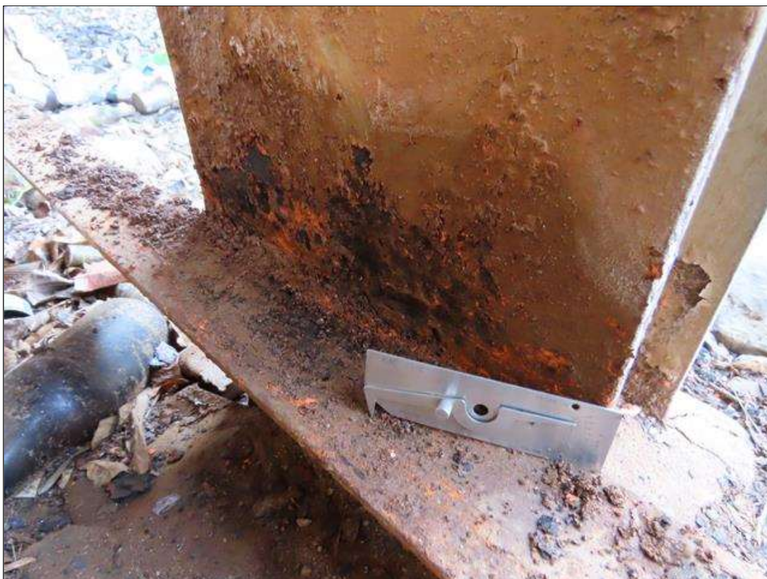
BENT 2 PILE 14 - NEAR FLANGE PITTING (UP TO 1/8IN PITTING, 5/16IN REMAIN) FOR 5IN W. X 3IN H. AT BOTTOM
