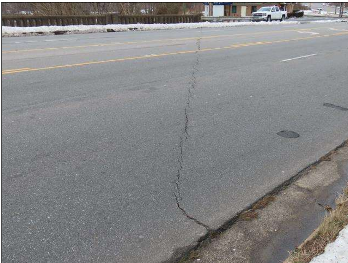
SPAN 1 AWS - FULL WIDTH TRANSVERSE CRACKING (UP TO 1/2IN) OVER END BENT 1 (SIMILAR OVER END BENT 2)
