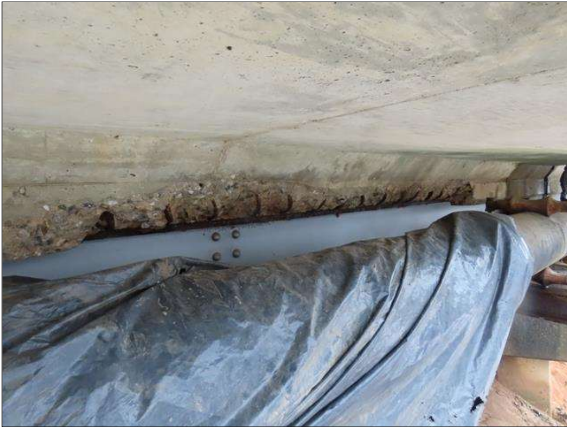
SPAN 1 DECK - SPALL & DELAMINATION (12FT L. X 1FT W. X 4IN D.) WITH EXPOSED REBAR RIGHT SIDE OF BEAM 11 HAUNCH AT FAR END (PAR PHOTO)
