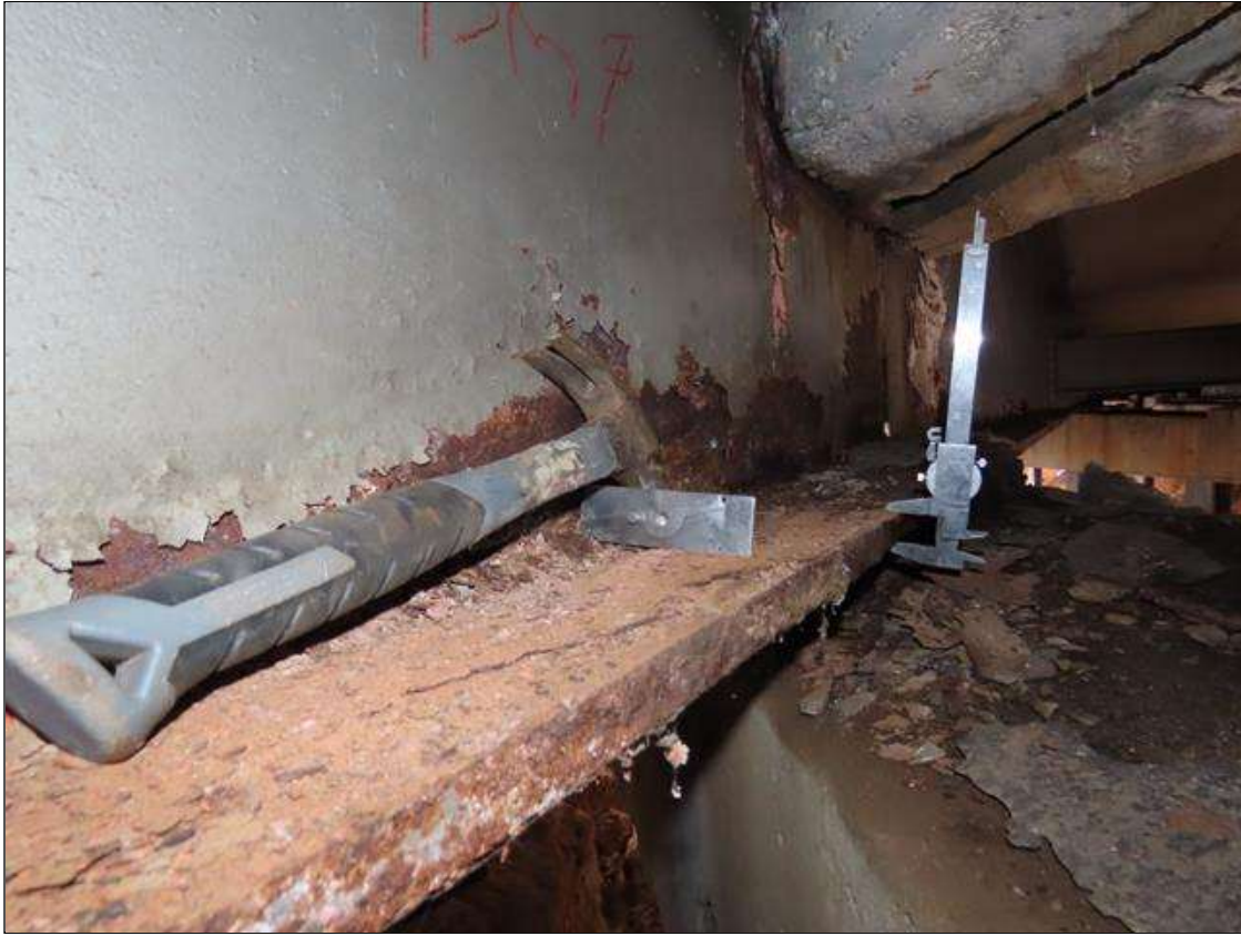
SPAN 5 BEAM 9 - BOTTOM FLANGE SECTION LOSS (UP TO 13% SL, 1/8IN SL, 13/16IN REMAIN) TO FULL WIDTH FOR 2FT L. & WEB SECTION LOSS (1/16IN SL, 9/16IN REMAIN) TO BOTTOM FOR 4IN H. X 3FT L. AT NEAR END
