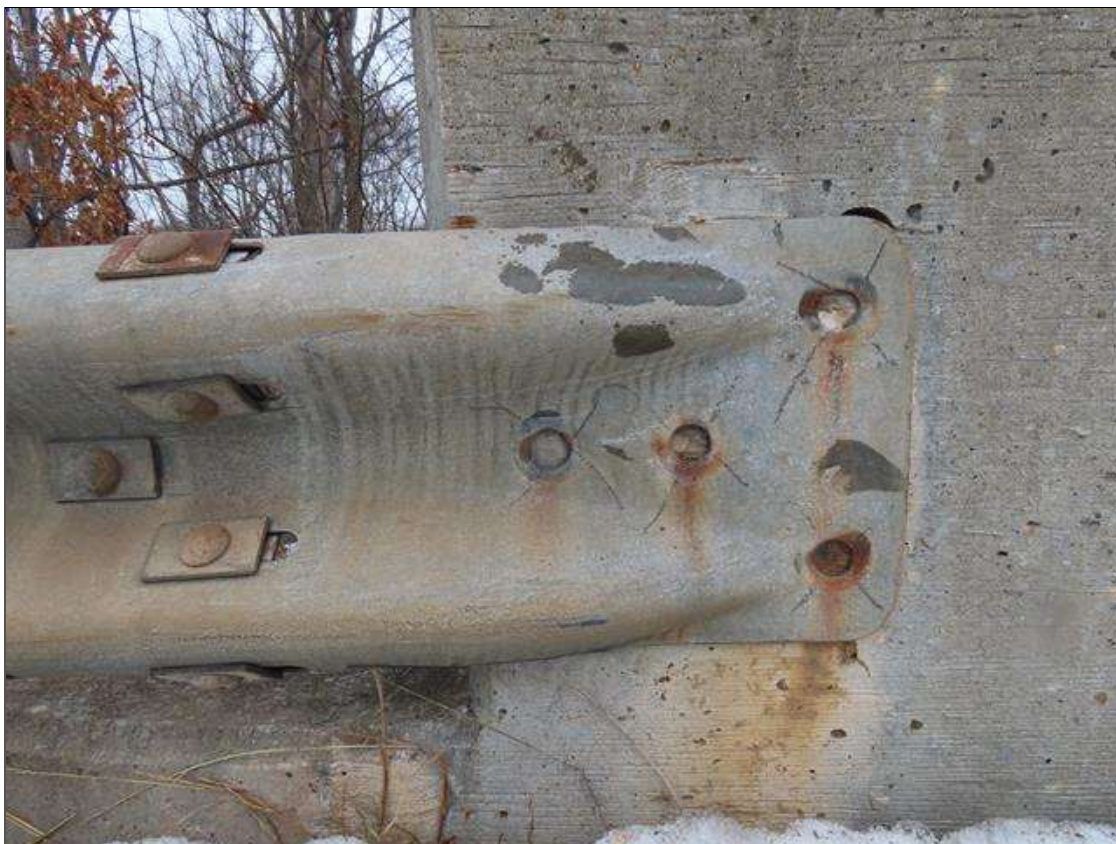
NEAR LEFT GUARDRAIL ATTACHMENT - NO ANCHOR BOLTS PRESENT (PAR PHOTO)
