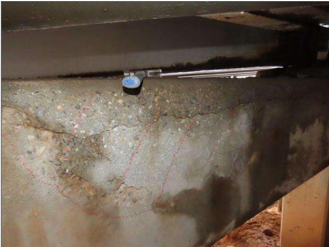
BENT 4 CAP - DELAMINATION (8 SQ. FT.) TO FAR FACE BELOW BAY 7
