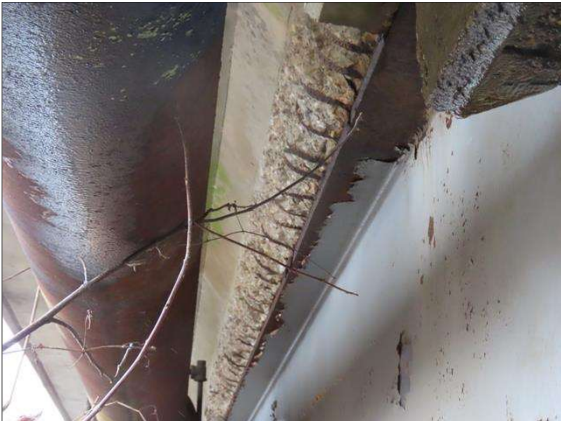
SPAN 4 DECK - SPALL (25FT X 6IN X 3IN) WITH EXPOSED REBAR TO RIGHT SIDE OF BEAM 11 HAUNCH AT FAR END (PAR PHOTO)
