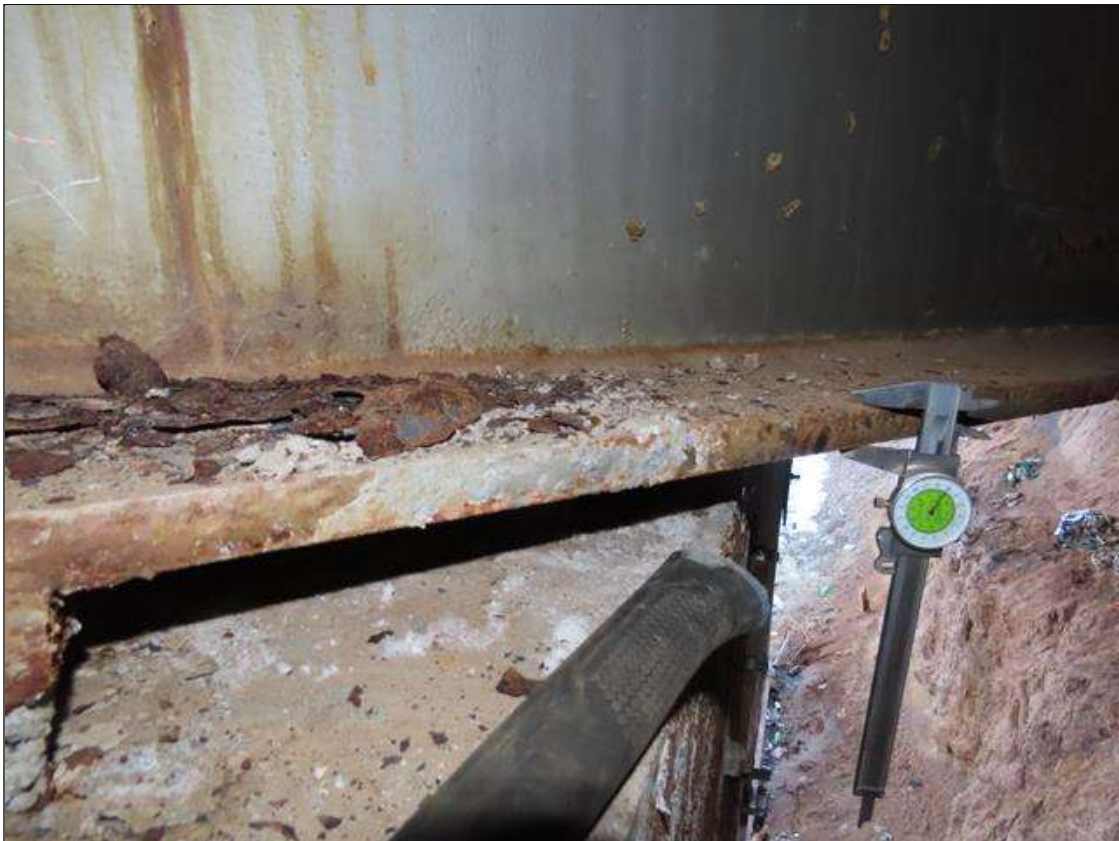
SPAN 2 BEAM 8 - BOTTOM FLANGE MODERATE SURFACE CORROSION FOR 2FT AT FAR END (SPAN 3 BEAM 8 SIMILAR FOR 1FT AT NEAR END)
