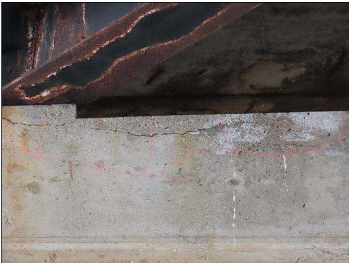
BENT 3 CAP - DELAMINATION (5FT X 1.5FT) TO NEAR FACE BELOW BEAM 7 & BAAY 7
