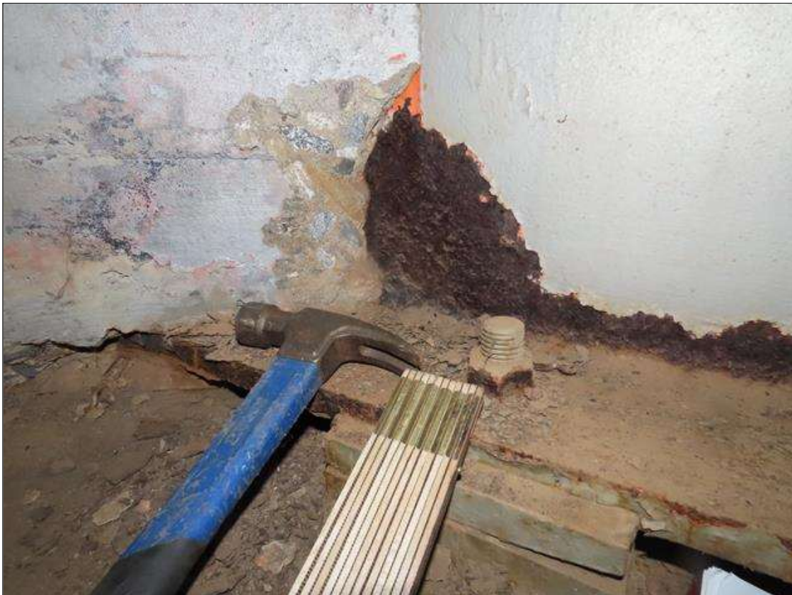
SPAN 1 BEAM 8 - WEB SECTION LOSS (1/16IN SL, 7/16IN REMAIN) TO RIGHT SIDE, 6IN X 6IN AT NEAR END BOTTOM
