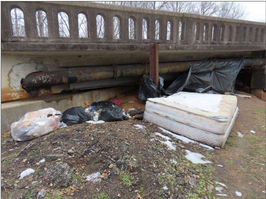
HEAVY DEBRIS & VAGRANT QUARTERS THROUGHOUT SPAN 1 OF BRIDGE, UNABLE TO OBTAIN FULL END BENT 1 PHOTO (PHOTO 1/2)
