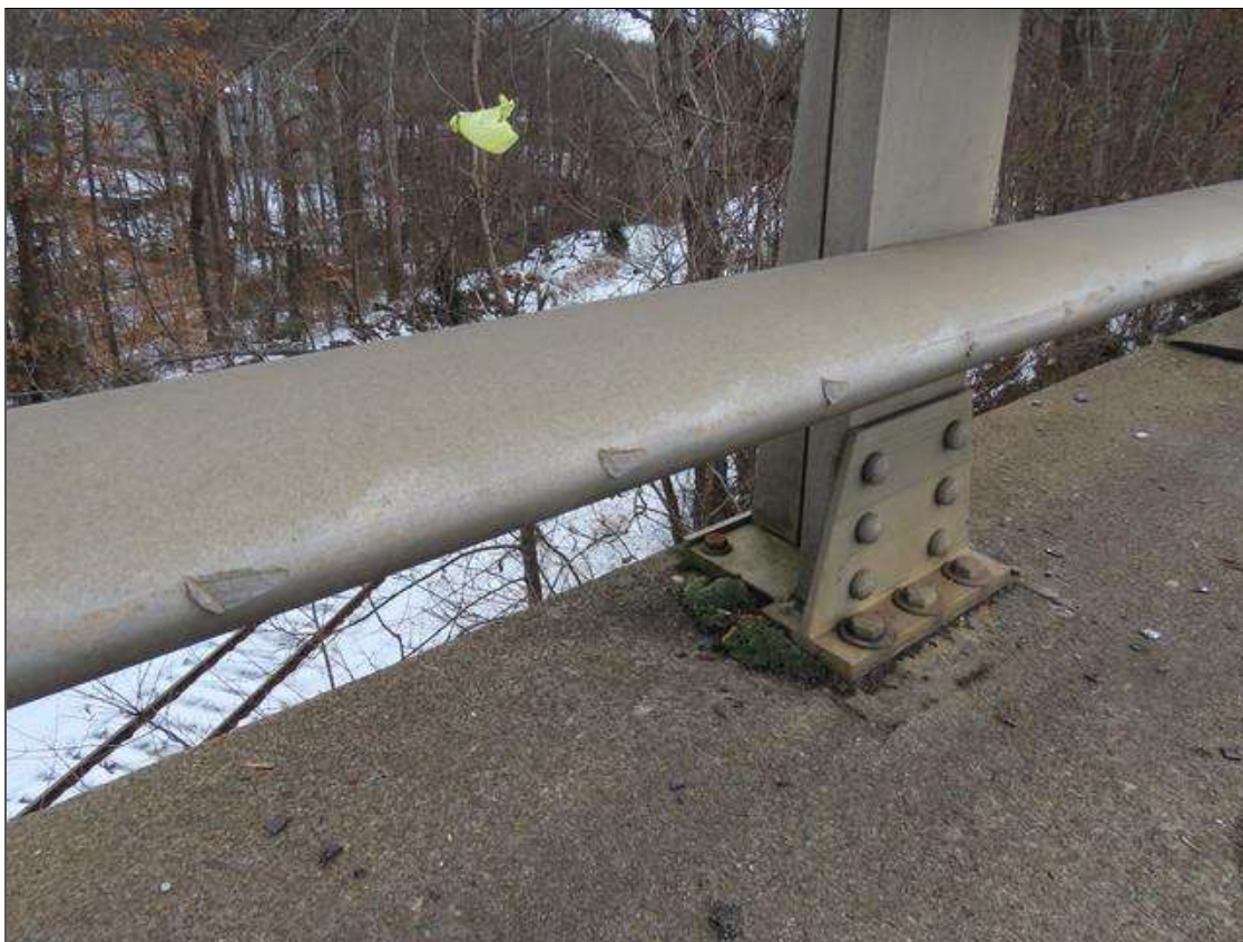
SPAN 4 LEFT RAIL - MINOR IMPACT DAMAGE (6FT L.) WITH MINOR GOUGING TO METAL RAILING AT FAR END
