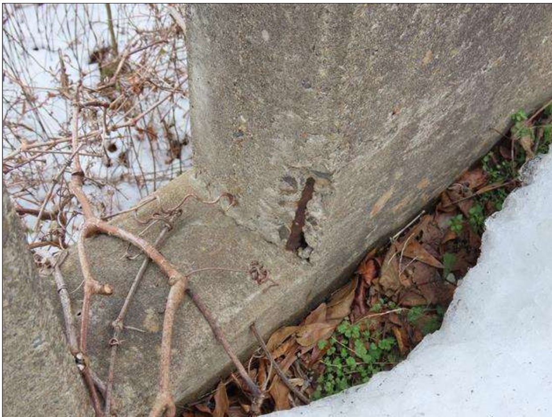
TYP. MINOR SPALLING (UP TO 6IN X 3IN X 1IN) WITH EXPOSED REBAR THROUGHOUT VERTICAL POSTS AT RIGHT RAIL, SPAN 5
