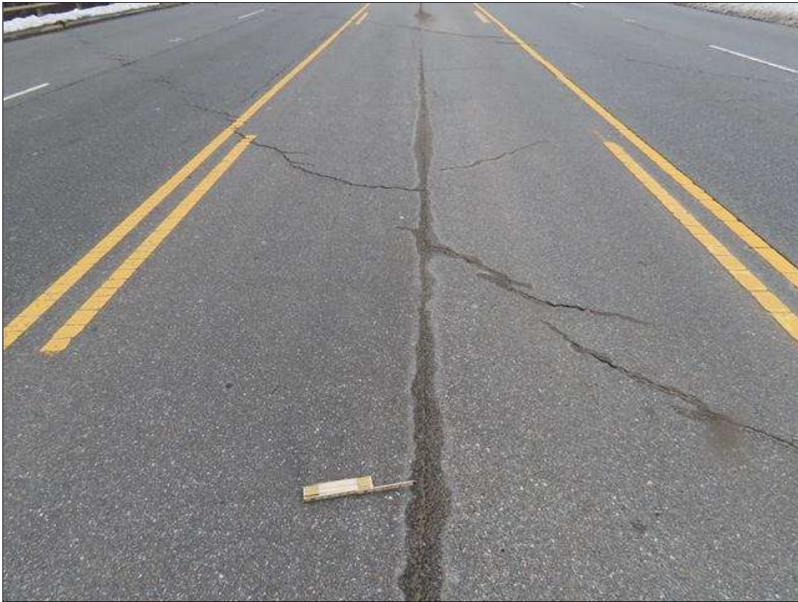
TYP. FULL LENGTH LONGITUDINAL CRACK (1/8IN) THROUGHOUT SPANS AT CENTER OF ROADWAY, SPAN 1
