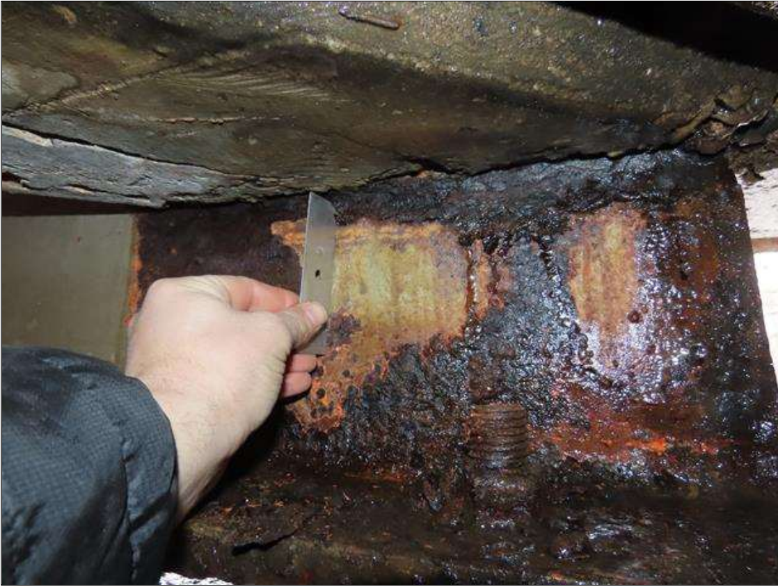
SPAN 2 BEAM 11 - WEB SECTION LOSS (3/8IN SL, 1/8IN REMAIN) FOR 18IN L. X 8IN H. AT NEAR END DIAPHRAGM (PAR PHOTO)
