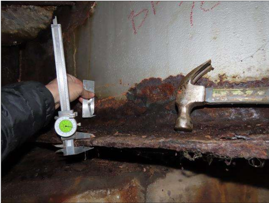
SPAN 5 BEAM 7 - BOTTOM FLANGE SECTION LOSS (UP TO 36% SL, 5/16IN SL, 9/16IN REMAIN) TO FULL WIDTH FOR 2FT L. & WEB SECTION LOSS (1/8IN SL, 7/16IN REMAIN) FOR 4FT L. AT NEAR END (PAR PHOTO)
