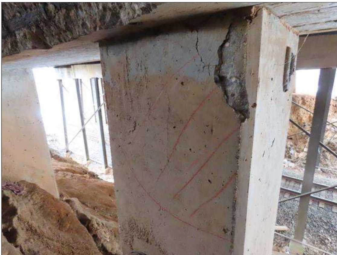
BENT 4 COLUMN 14 - SPALL & DELAMINATION (FULL WIDTH X 2FT X UP TO 1IN) TO FAR FACE AT TOP
