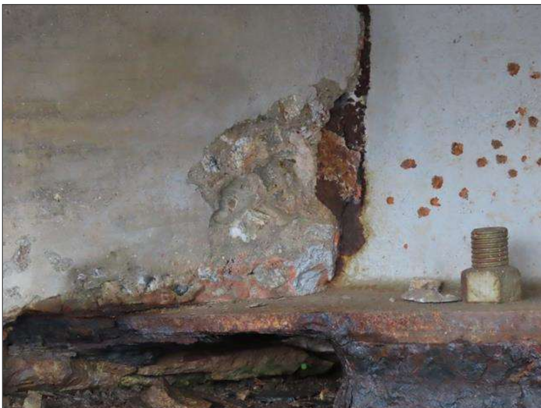
TYP. INTERMITTENT SPALLING (UP TO 8IN X 2IN X 1IN) WITH NO EXPOSED REBAR TO BACKWALL AT BOTTOM FLANGE ENDS, RIGHT OF BEAM 11
