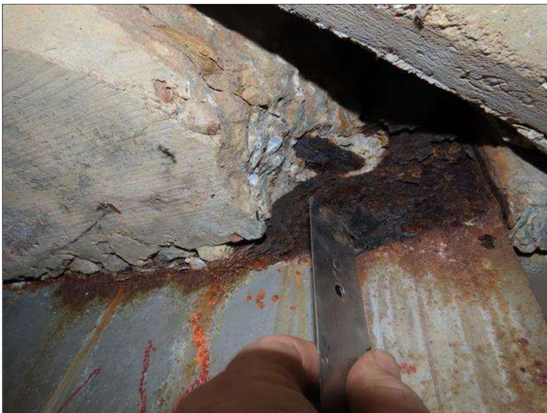
SPAN 4 BEAM 8 - WEB SECTION LOSS (1/16IN SL, 9/16IN REMAIN) FOR 8IN L. X 3IN H. AT FAR END DIAPHRAGM
