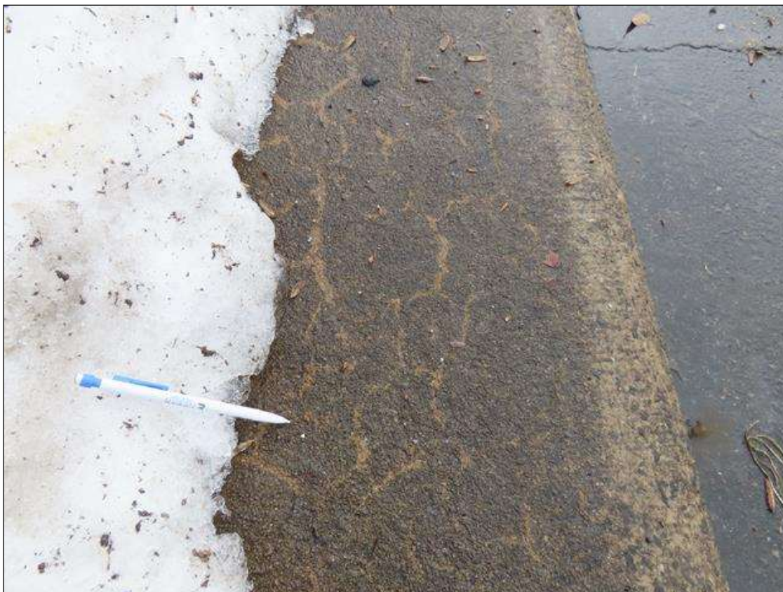
TYP. HAIRLINE MAP CRACKING THROUGHOUT LEFT SIDE SIDEWALK, SPAN 1
