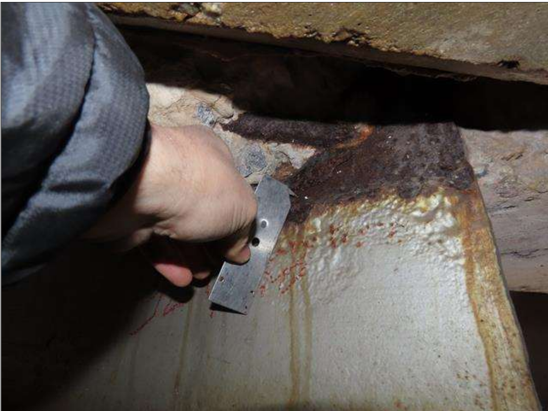
SPAN 2 BEAM 8 - WEB SECTION LOSS (1/4IN SL, 1/4IN REMAIN) FOR 16IN L. X 3IN H. AT NEAR END DIAPHRAGM (PAR PHOTO)
