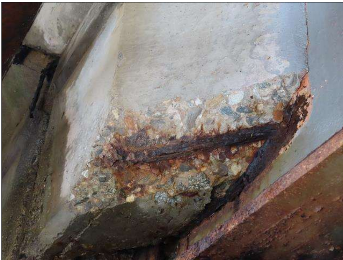
SPAN 2 RIGHT OVERHANG DIAPHRAGM AT NEAR END - SPALL (12IN X 8IN X 2IN) WITH EXPOSED REBAR TO FAR BOTTOM CORNER (PAR PHOTO)
