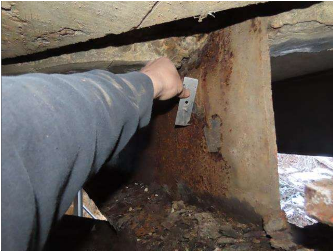
SPAN 3 BEAM 9 - WEB SECTION LOSS (3/8IN SL, 1/4IN REMAIN) TO FULL HEIGHT X 2FT L. AT NEAR END DIAPHRAGM (PAR PHOTO)
