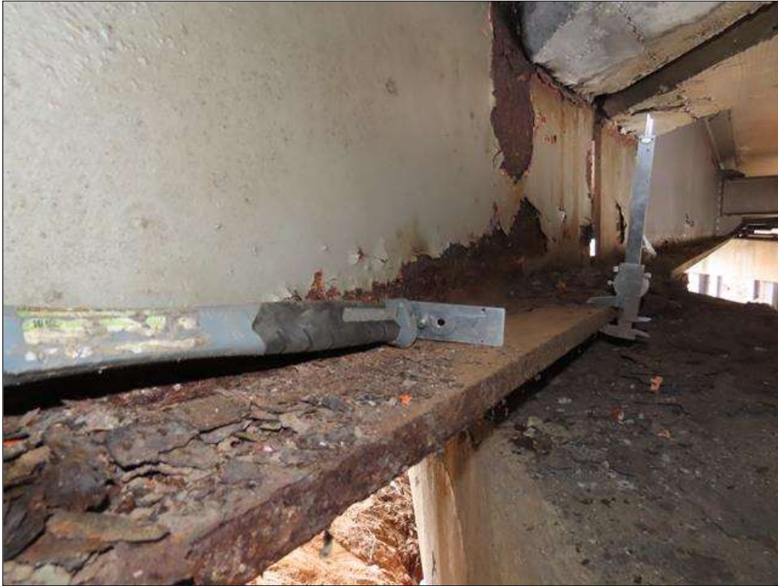
SPAN 5 BEAM 10 - BOTTOM FLANGE SECTION LOSS (UP TO 7% SL, 1/16IN SL, 7/8IN REMAIN) TO FULL WIDTH FOR 2FT L. & WEB SECTION LOSS (1/16IN SL, 9/16IN REMAIN) X 3IN H. FOR 2FT L. AT NEAR END
