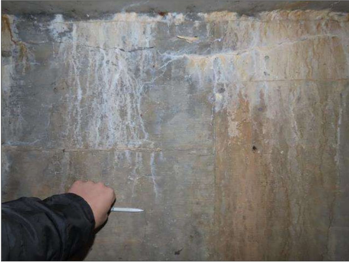
TYP. INTERMITTENT VERTICAL & TRANSVERSE HAIRLINE CRACKING THROUGHOUT END BENT 2 BACKWALL BAY 5
