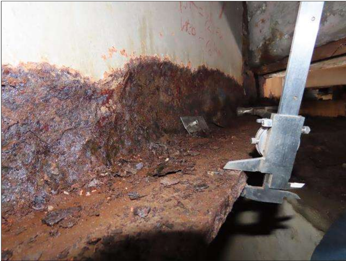
SPAN 1 BEAM 7 - BOTTOM FLANGE SECTION LOSS (UP TO 33% SL, 1/4IN SL, 1/12IN REMAIN) TO FULL WIDTH & WEB SECTION LOSS (3/8IN SL, AVG. 1/8IN REMAIN) X 6IN H. FOR 10FT L. AT FAR END (PAR PHOTO)
