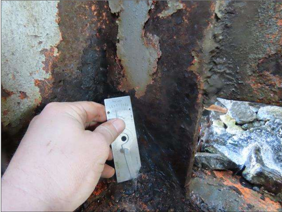
BENT 3 PILE 17 - NEAR FLANGE SECTION LOSS (UP TO 1/8IN SL, 5/16IN REMAIN) FOR 6IN W. X 6IN H. AT BOTTOM (FAR FLANGE SIMILAR, 1/16IN PITTING)
