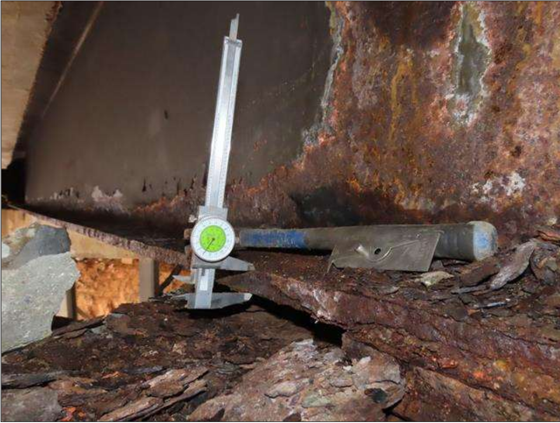
SPAN 3 BEAM 7 - BOTTOM FLANGE SECTION LOSS (UP TO 7% SL, 1/16IN SL, 13/16IN REMAIN) TO FULL WIDTH FOR 10FT L. & WEB SECTION LOSS (1/8IN SL, 7/16IN REMAIN) X 3IN H. FOR 5FT L. AT FAR END
