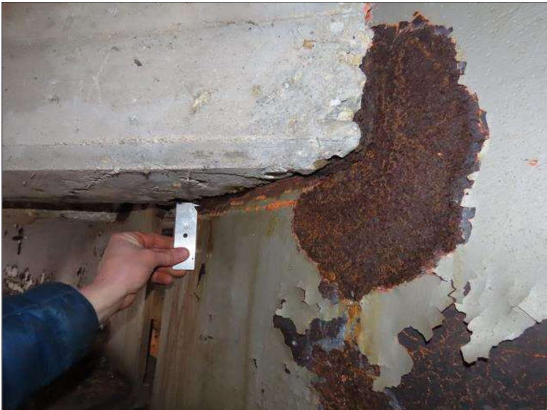
SPAN 5 BEAM 10 - WEB SECTION LOSS (1/4IN SL, 3/8IN REMAIN) FOR 20IN L. X 6IN H. AT NEAR END DIAPHRAGM (PAR PHOTO)
