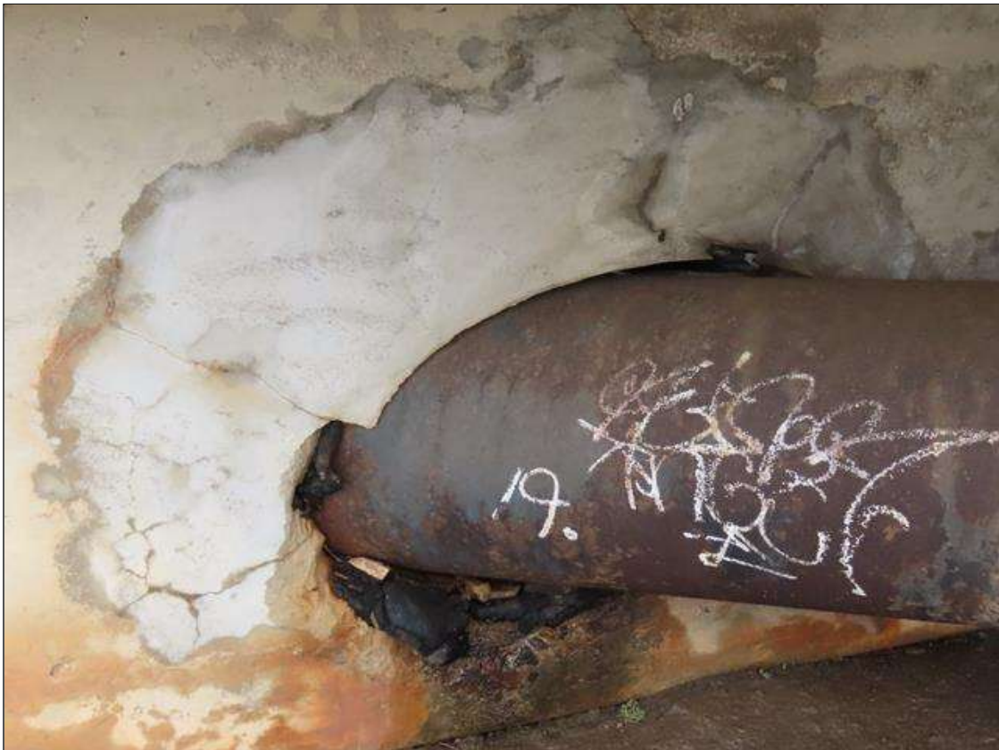
END BENT 1 ABUTMENT - HAIRLINE MAP CRACKING (4 SQ. FT.) THROUGHOUT RIGHT SIDE UTILITY OPENING PATCH
