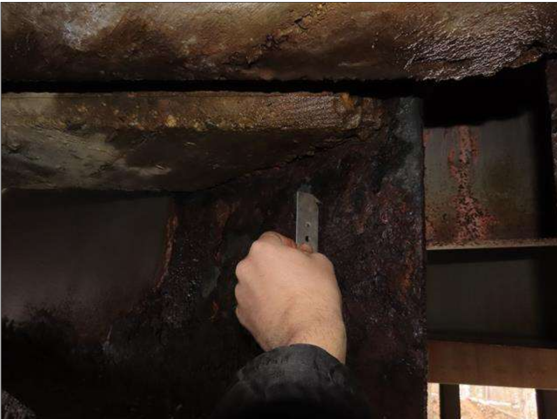
SPAN 4 BEAM 7 - WEB SECTION LOSS (1/16IN SL, 1/2IN REMAIN) FOR 20IN L. X 20IN H. AT FAR END DIAPHRAGM
