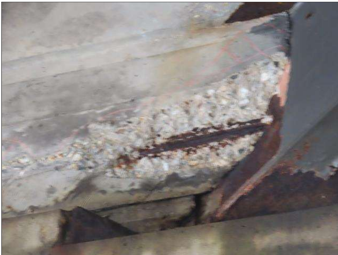
SPAN 3 BAY 9 NEAR DIAPHRAGM - SPALL (24IN X 24IN X 5IN) WITH EXPOSED REBAR ADJACENT TO BEAM 9 (PAR PHOTO)
