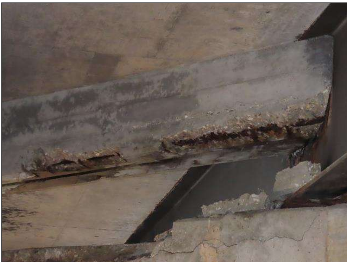
SPAN 4 BAY 7 NEAR DIAPHRAGM - 2X SPALLS (UP TO 40IN X 8IN X 4IN) WITH EXPOSED REBAR THROUGHOUT (PAR PHOTO)
