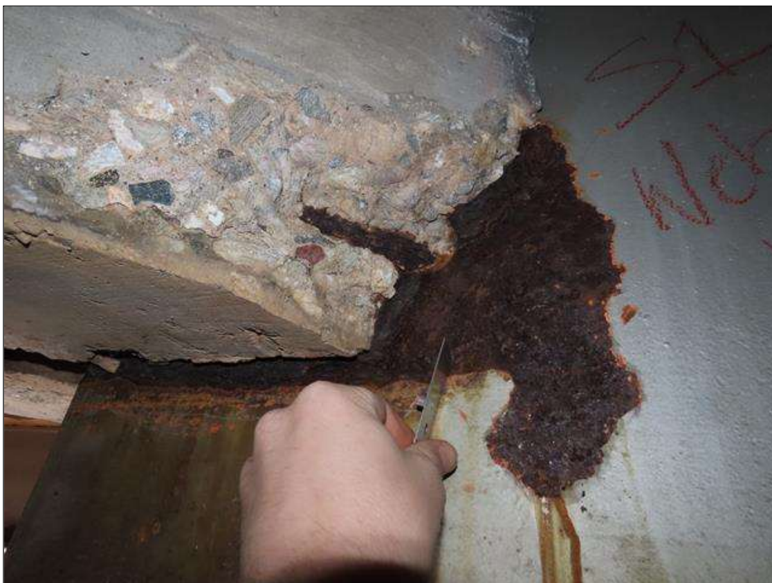
SPAN 1 BEAM 10 - WEB SECTION LOSS (1/4IN SL, 1/4IN REMAIN) FOR 16IN L. X 8IN H. AT FAR END DIAPHRAGM (PAR PHOTO)
