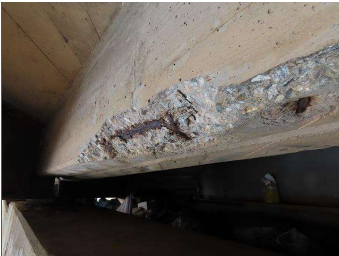
SPAN 2 BAY 9 NEAR DIAPHRAGM - SPALL (40IN X 12IN X 4IN) WITH EXPOSED REBAR THROUGHOUT (PAR PHOTO)
