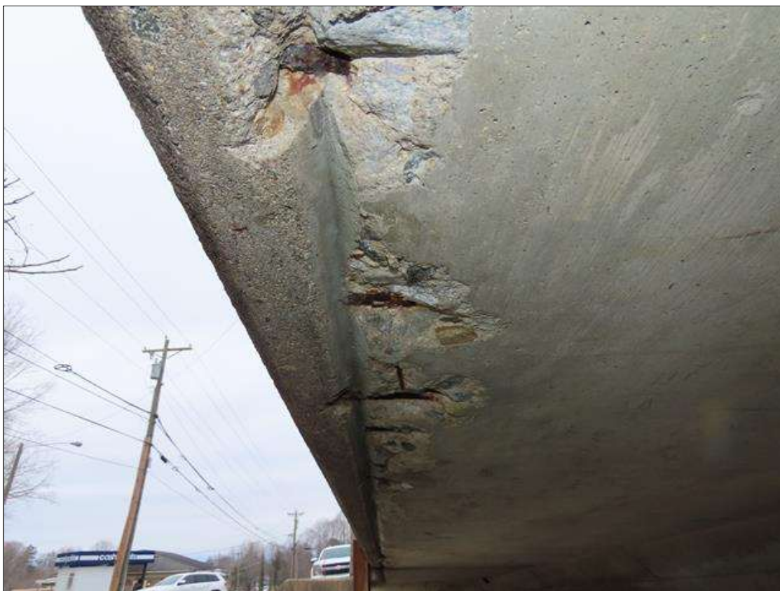
TYP. MINOR SPALLING (UP TO 6IN DIA. X 1IN D.) WITH EXPOSED REBAR THROUGHOUT RIGHT SIDE DRIP LINE, SPAN 1 RIGHT OVERHANG
