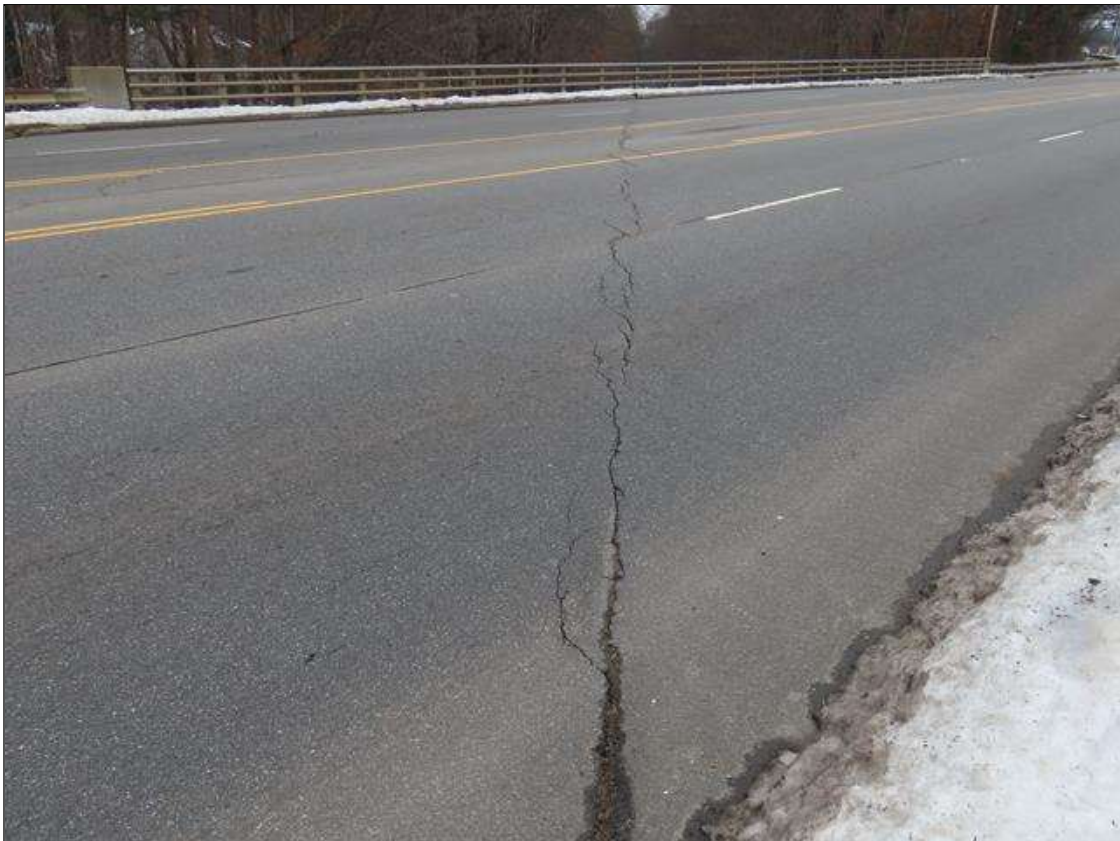
SPAN 2 AWS - FULL WIDTH TRANSVERSE CRACK (UP TO 1/4IN) OVER BENT 2 (SIMILAR OVER ALL INTERIOR BENTS)
