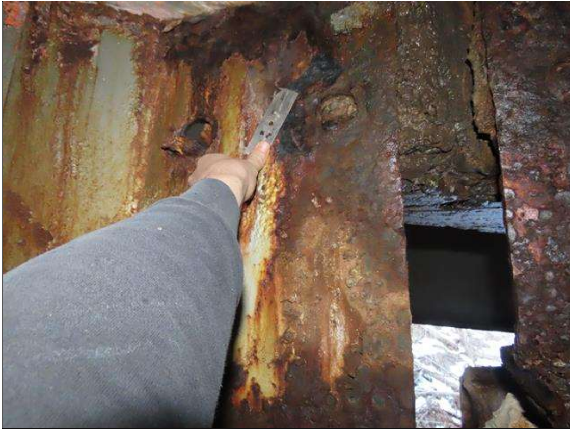
SPAN 3 BEAM 7 - WEB SECTION LOSS (1/8IN SL, 7/16IN REMAIN) FOR 18IN L. X 12IN H. AT NEAR END DIAPHRAGM
