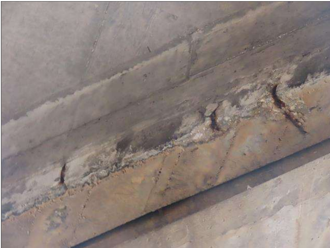
TYP. MULTIPLE MINOR SPALLS (UP TO 8IN X 3IN X 1/2IN) WITH EXPOSED REBAR THROUGHOUT SPAN 3 NEAR & FAR DIAPHRAGMS, SPAN 3 BAY 9 FAR DIAPHRAGM
