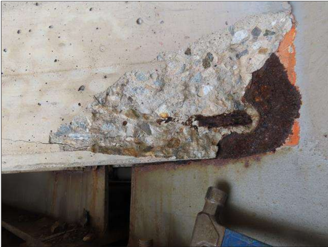
SPAN 2 BAY 10 NEAR DIAPHRAGM - SPALL (12IN X 8IN X 2IN) WITH EXPOSED REBAR ADJACENT TO BEAM 10 (PAR PHOTO)
