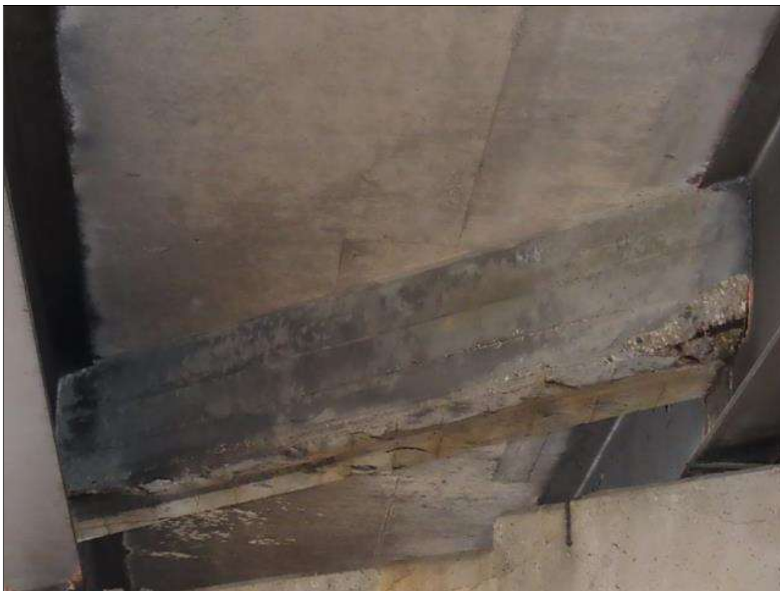
SPAN 4 BAY 8 NEAR DIAPHRAGM - SPALL & DELAMINATION (UP TO 48IN X 8IN X 2IN) WITH EXPOSED REBAR THROUGHOUT (PAR PHOTO)
