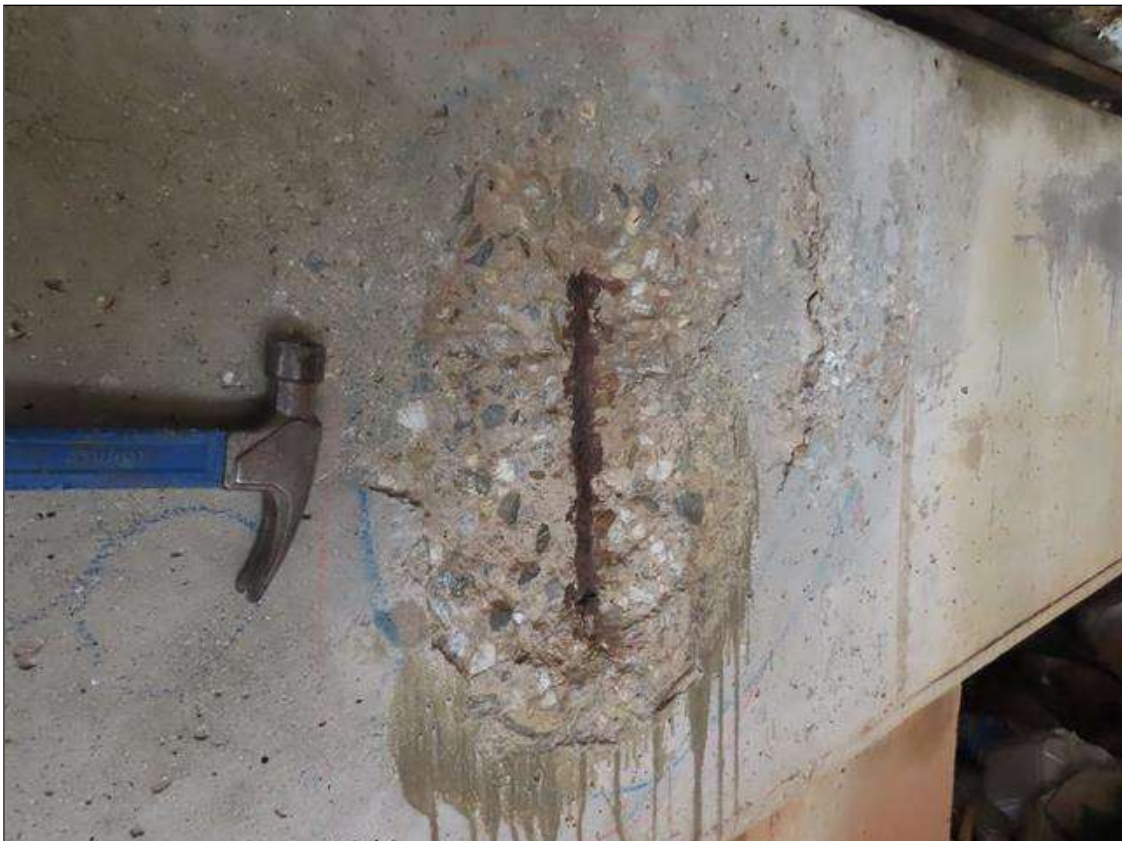
BENT 1 CAP - SPALL (24IN X 16IN X 1IN) WITH EXPOSED REBAR TO FAR FACE BELOW BEAM 8
