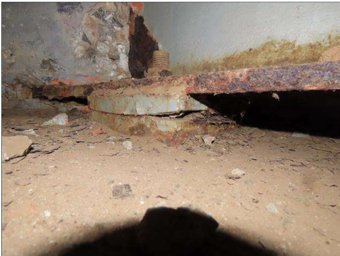
TYP. MINOR SURFACE CORROSION TO BEARINGS AT END BENT 1, BEAM 7 (BEAM 8-10 SIMILAR)
