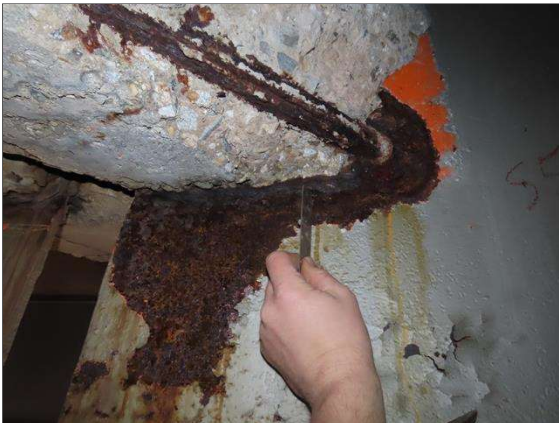
SPAN 5 BEAM 9 - WEB SECTION LOSS (5/16IN SL, 5/16IN REMAIN) FOR 16IN L. X 9IN H. AT NEAR END DIAPHRAGM (PAR PHOTO)
