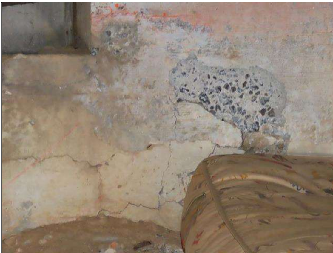
END BENT 1 CAP - SPALL & DELAMINATION (3.5FT X 1.5FT X 1IN) WITH NO EXPOSED REBAR TO FACE BELOW BAY 7
