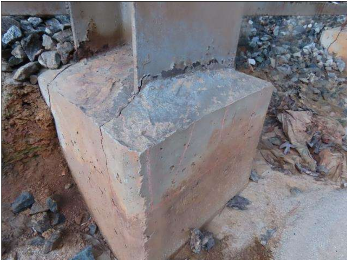
TYP. DELAMINATION (FULL WIDTH X 1FT H.) THROUGHOUT FACES OF CONCRETE AT BASE OF COLUMNS, BENT 3 PILE 15
