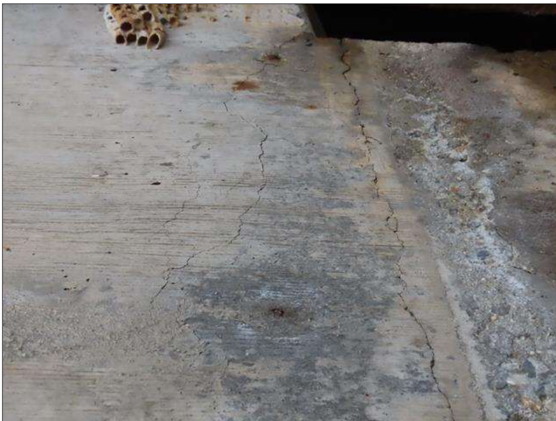
BENT 4 CAP - VERTICAL HAIRLINE TO 1/32IN CRACKING (FULL HEIGHT) TO NEAR FACE BELOW BAY 6
