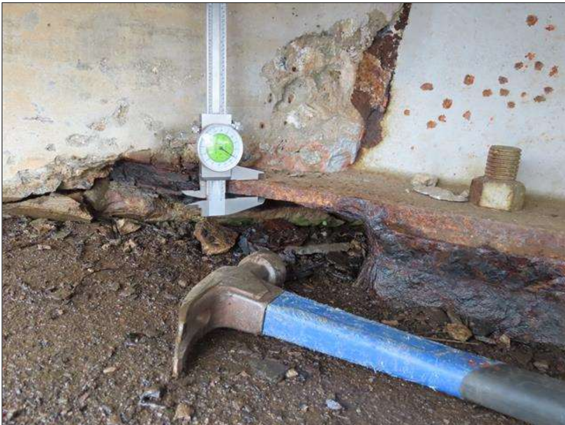
SPAN 1 BEAM 11 - BOTTOM FLANGE SECTION LOSS (13% SL, 3/16IN SL, 9/16IN REMAIN) TO RIGHT SIDE, 3IN W. FOR 6IN L. AT NEAR END BEHIND BEARING
