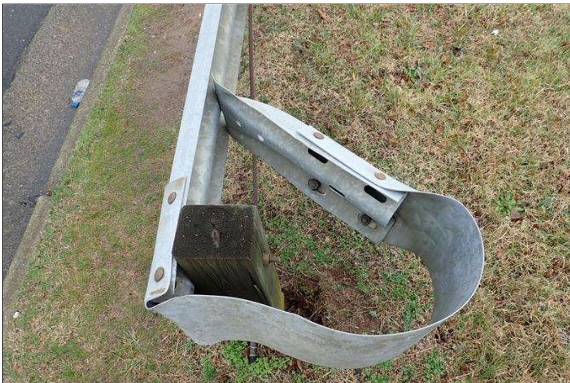
(PAR) southwest guardrail termination, impact damage (3')
