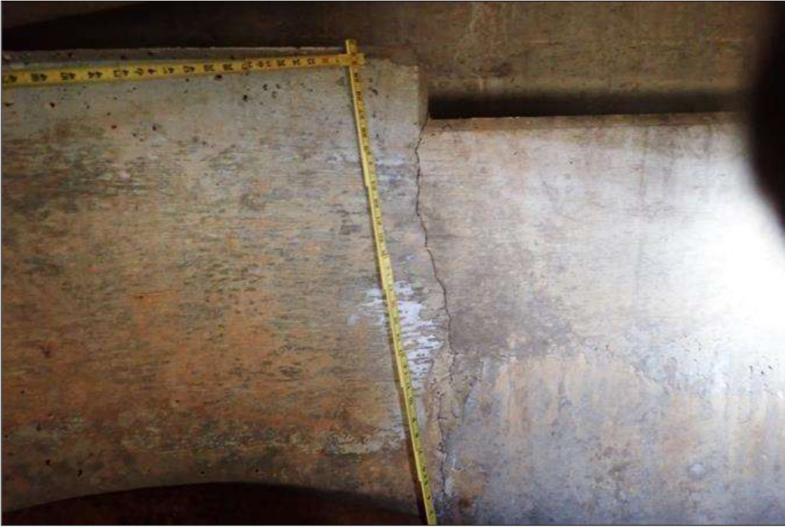
End Bent 2 Cap 1: at beam 5, vertical crack (1/16" x 2') at cold joint
