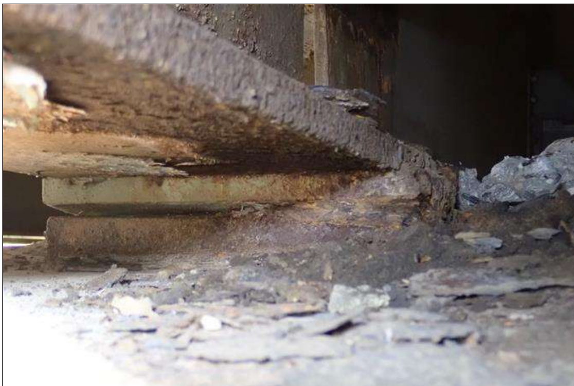
Span 2 Beam 9 Near Bearing 9: pack rust
