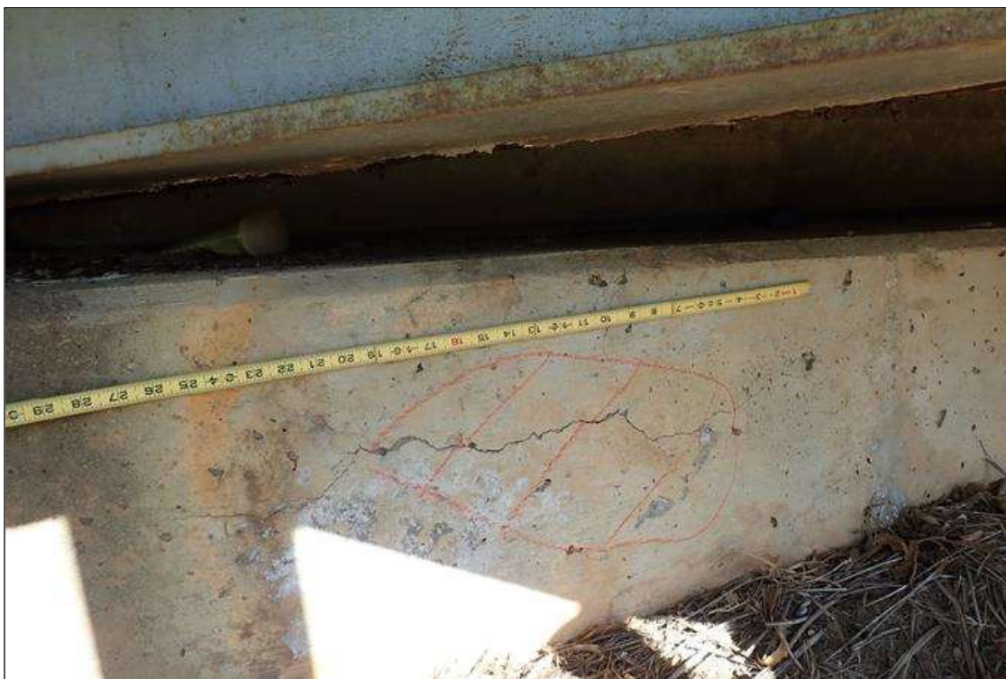
End Bent 1 Cap 1: face of cap, below beam 11, longitudinal crack (1/16" x 2') with delamination (16" x 10")
