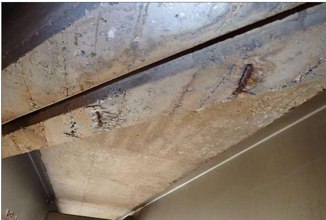
Span 4 Deck: bent 4 end diaphragm, bay 7, underside, multiple spalls (up to 8" x 6" x 1"); similar bays 8, 9 and 10
