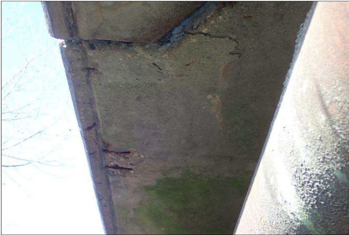
Span 4 Deck: underside of right overhang at bent 4, (2) spalls (8" diameter x 1") with exposed rusted rebar
