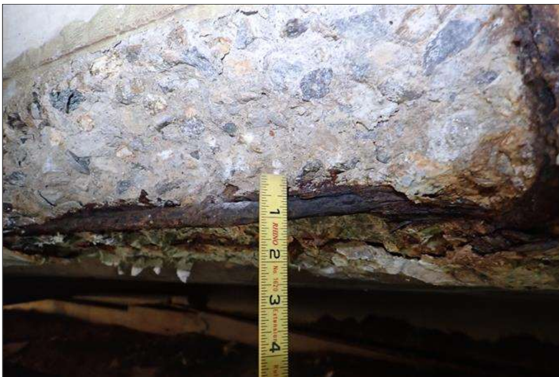
Span 2 Deck: (PAR) bent 1 end diaphragm, bay 7, failed previous repair (10' x 10" x 4") with section loss on rebar (3/8" remaining)
