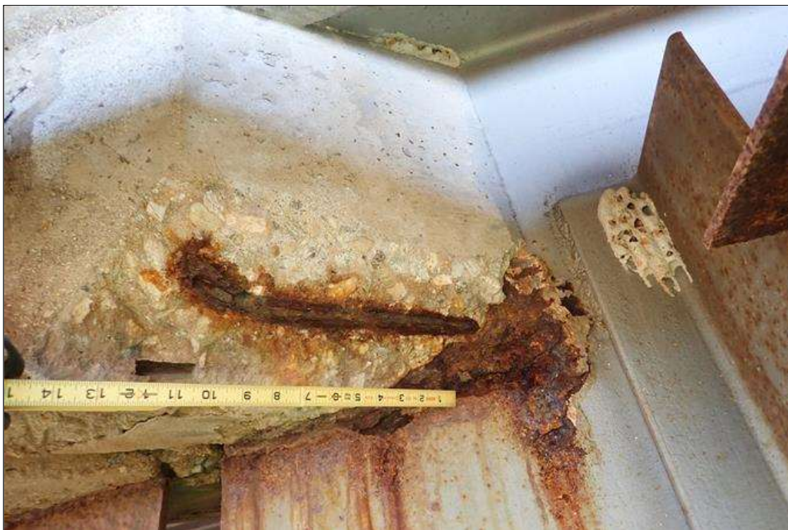
Span 5 Deck: bent 4 end diaphragm, right overhang, spall (12" x 6" x 2") with exposed rusted rebar
