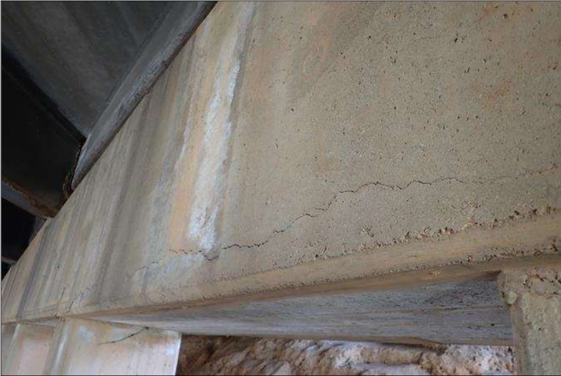
Bent 4 Cap 1: (PAR) span 5 face, from beam 8 to 11, longitudinal cracks (1/8" x 30') at top and bottom corners with delamination (up to full height x 30') and spalls (19' x up to 20" x 2") with exposed rusted rebar; cracks and delamination similar on span 4 face
