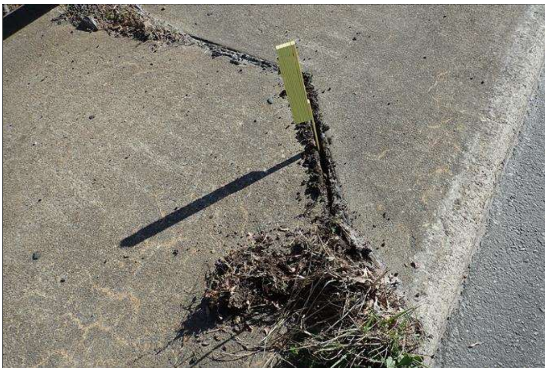
Bent 1 Joint : left sidewalk, joint material separated with debris and vegetation
