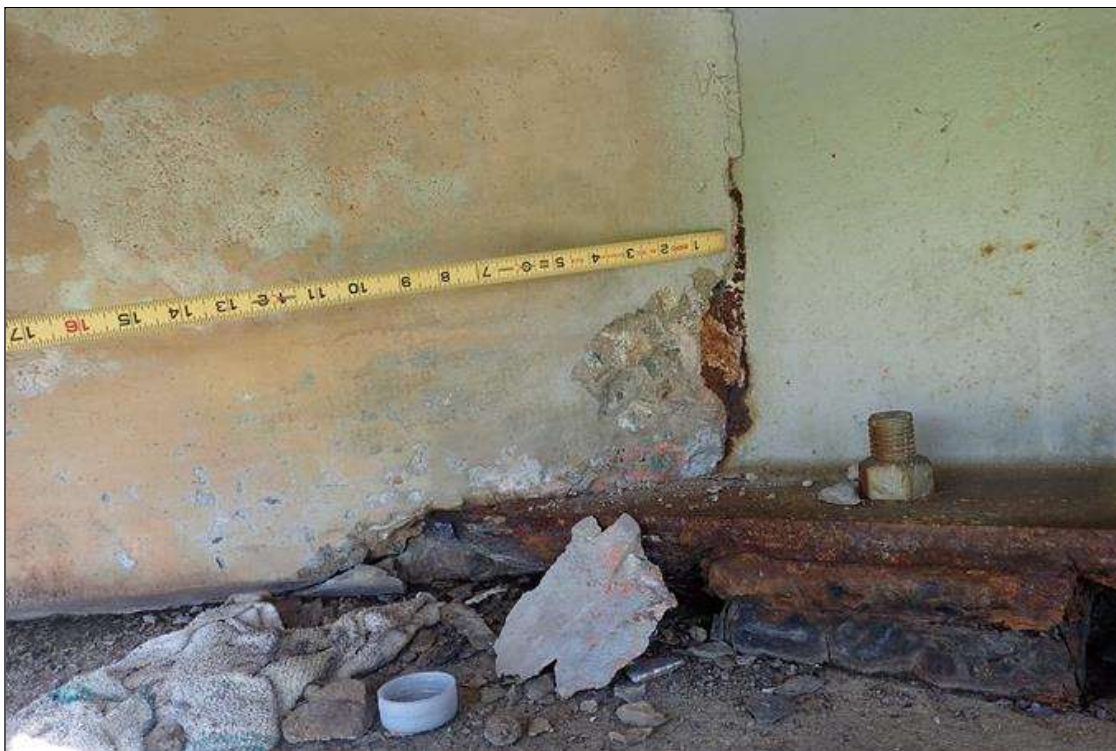
End Bent 1 Abutment/Backwall : right side of beam 11, bottom flange, spall (5" x 3" x 1/2")
