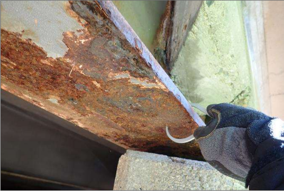
Span 1 Beam 11: (PAR) at bent 1, corrosion with section loss: bottom flange, (0.6" average remaining x 3'); web at end diaphragm, (1/8" remaining x 3" wide x 19")
