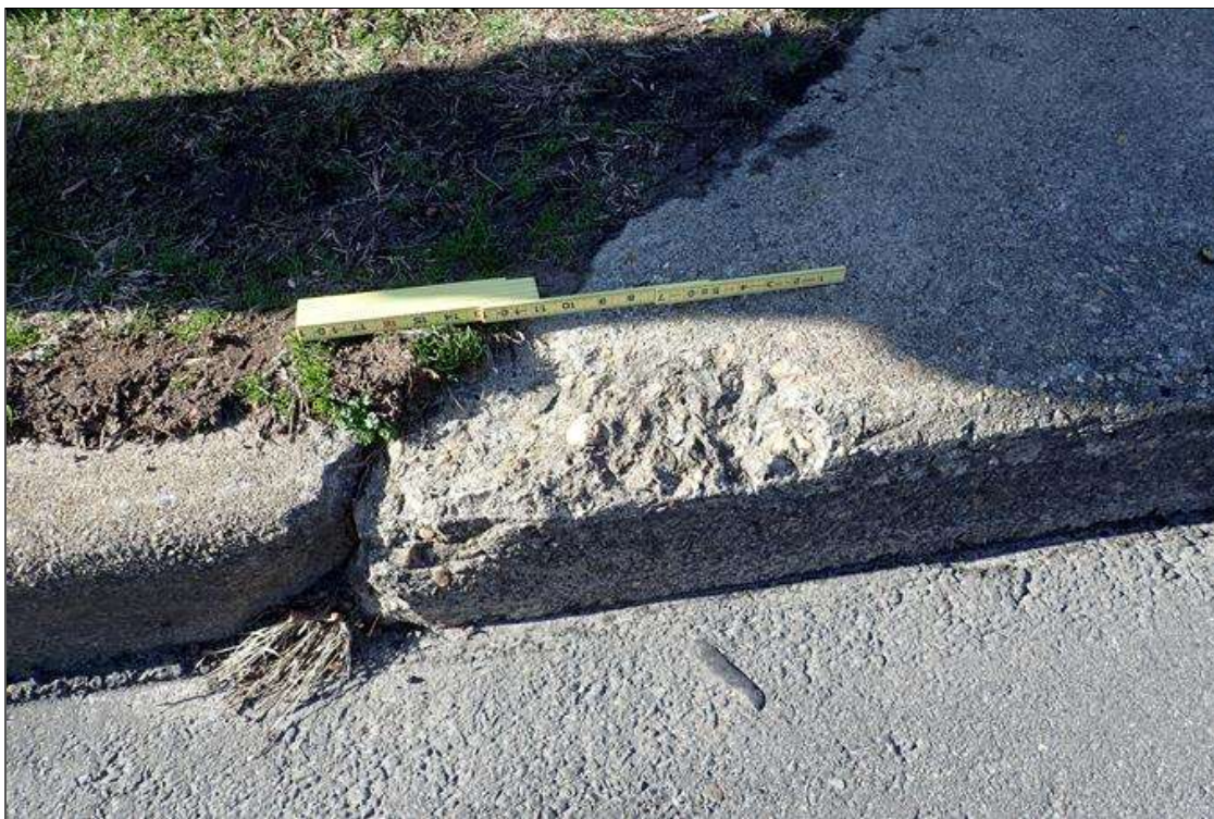
Span 5 Right Bridge Rail: at end bent 2, corner of sidewalk, spall (16" x 5" x 1.5")
