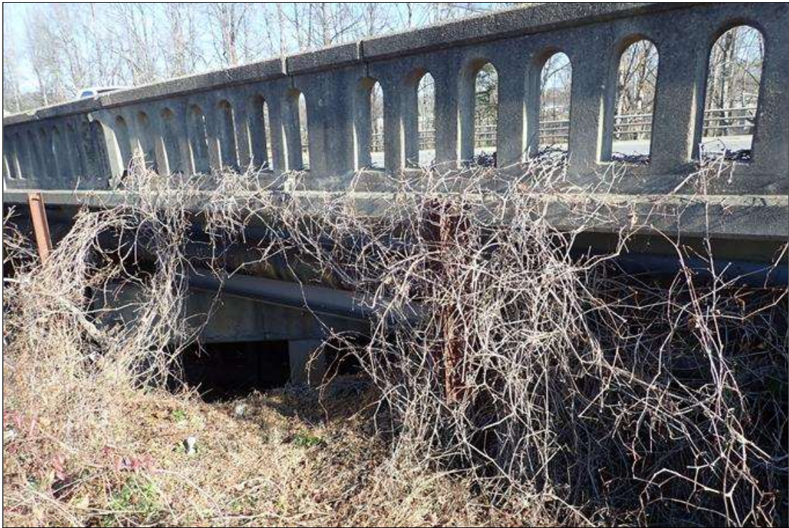
Span 5 Deck: right edge of deck, vegetation (15')
