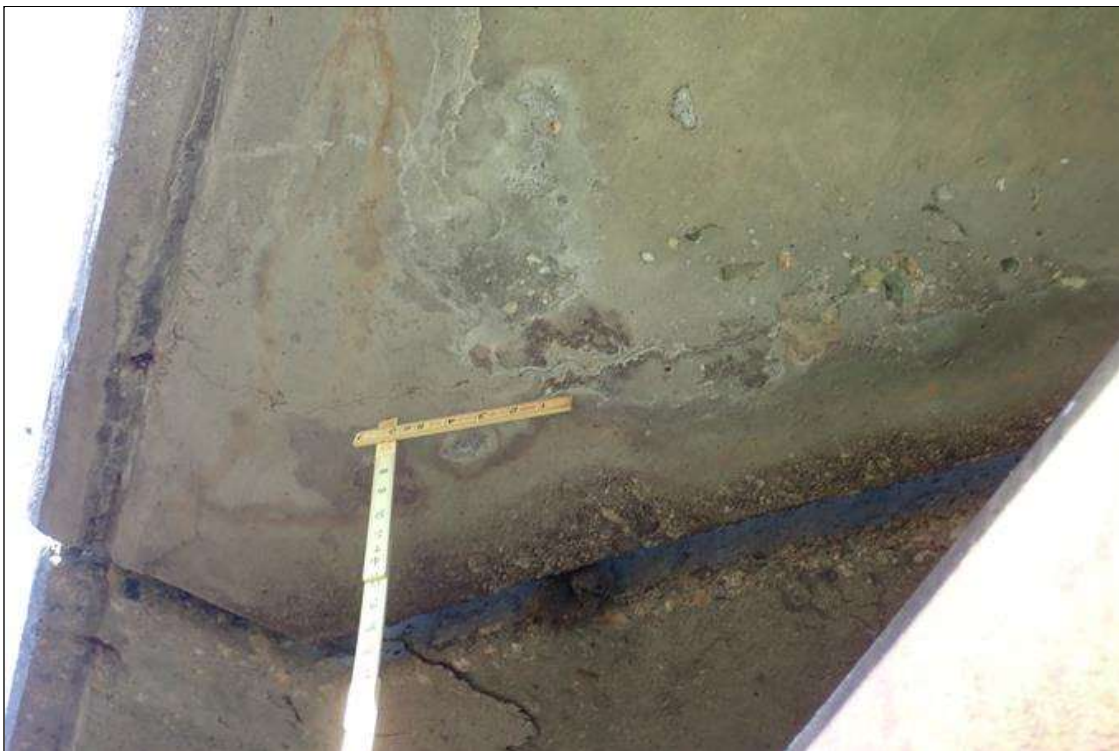
Span 5 Deck: underside of right overhang at bent 4, transverse crack (1/32" x 3')
