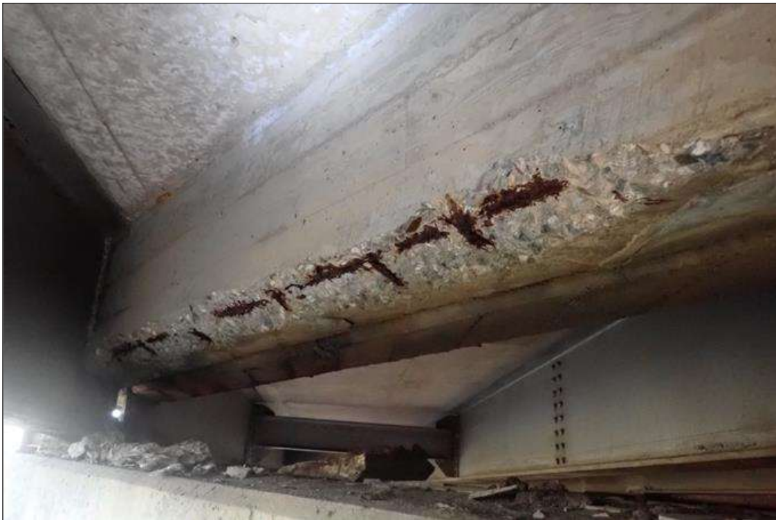
Span 2 Deck: bent 1 end diaphragm, bay 10, at beam 11, spall (6' x 7" x 2") with exposed rusted rebar
