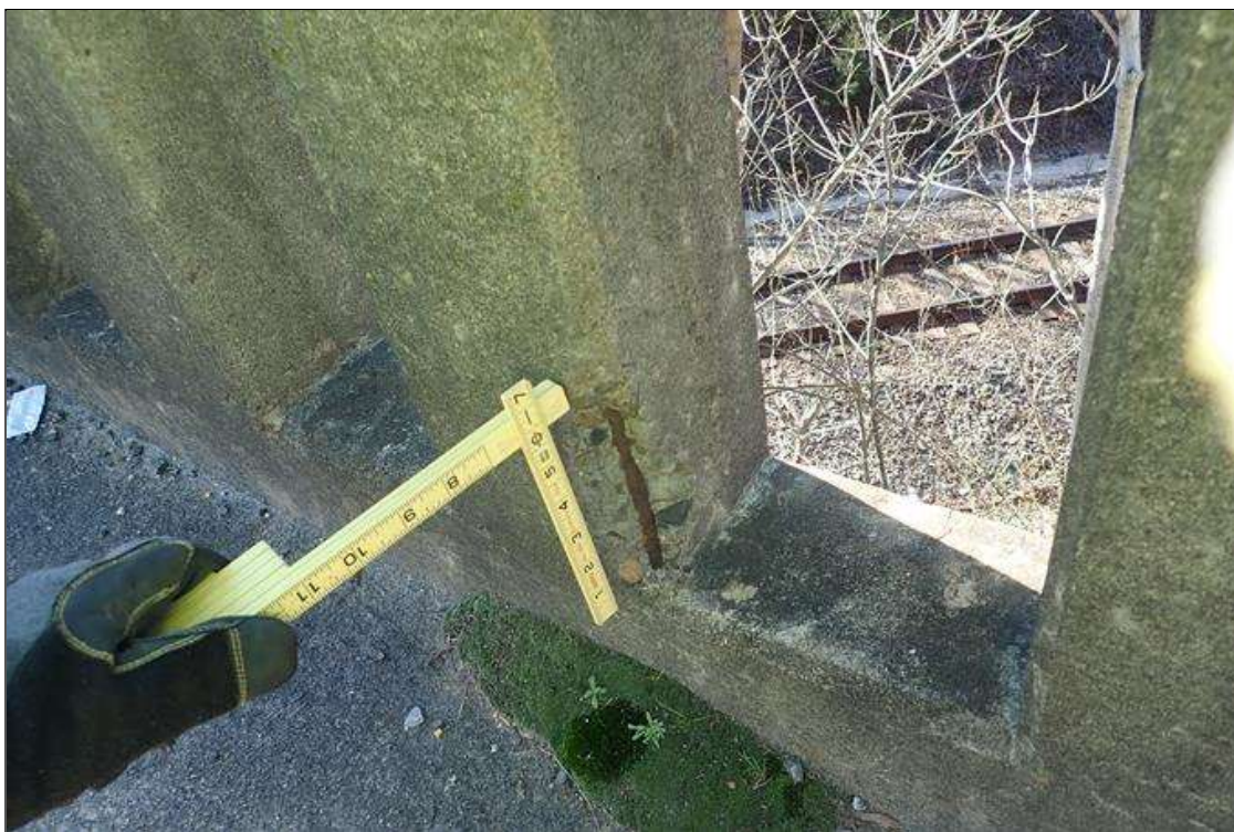
Span 1 Right Bridge Rail: rail posts at random, (6) spalls (up to 6" x 2" x 1") with exposed rusted rebar
