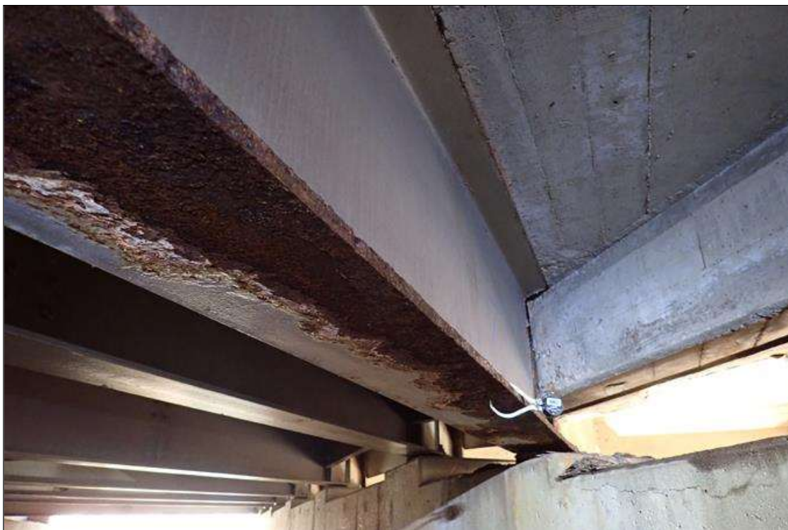
Span 1 Beam 7: (PAR) at bent 1, bottom flange, corrosion with section loss (0.6" average remaining x 11')
