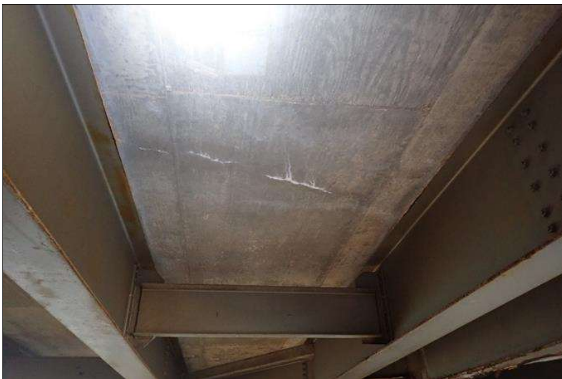
Span 2 Deck: underside, bay 5, at midspan, transverse crack (hairline x 7') with efflorescence
