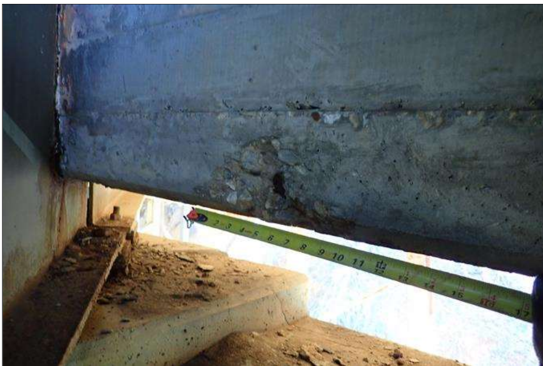
Span 1 Deck: bent 1 end diaphragm, bay 9 at beam 9, spall (12" x 4" x 1") with exposed rusted rebar
