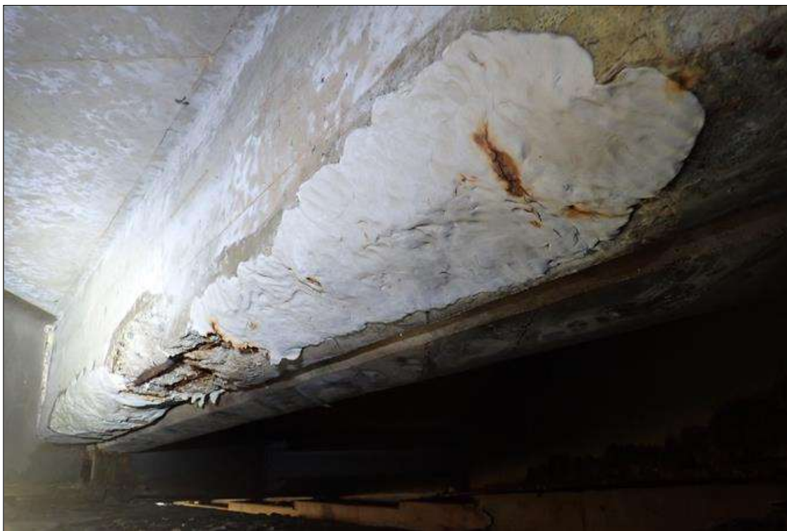
Span 2 Deck: (PAR) bent 1 end diaphragm, bay 7, failed previous repair (10' x 10" x 4") with section loss on rebar (3/8" remaining)
