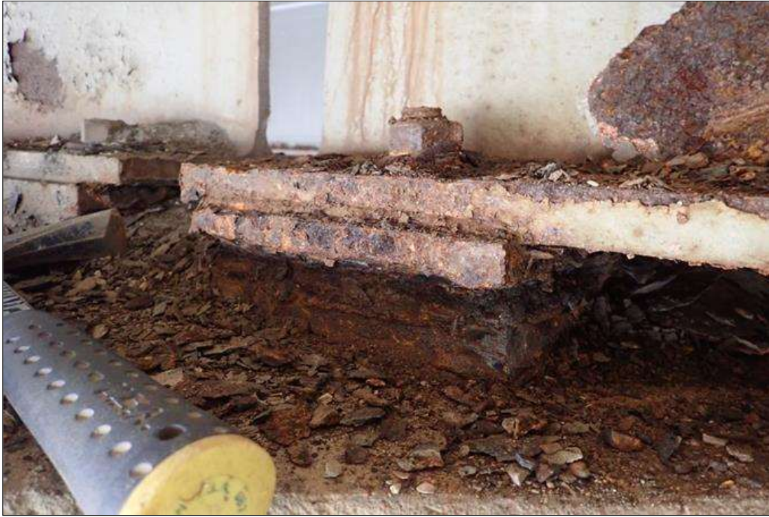
Span 5 Beam 10 Near Bearing 10: (PAR) bearing frozen with pack rust
