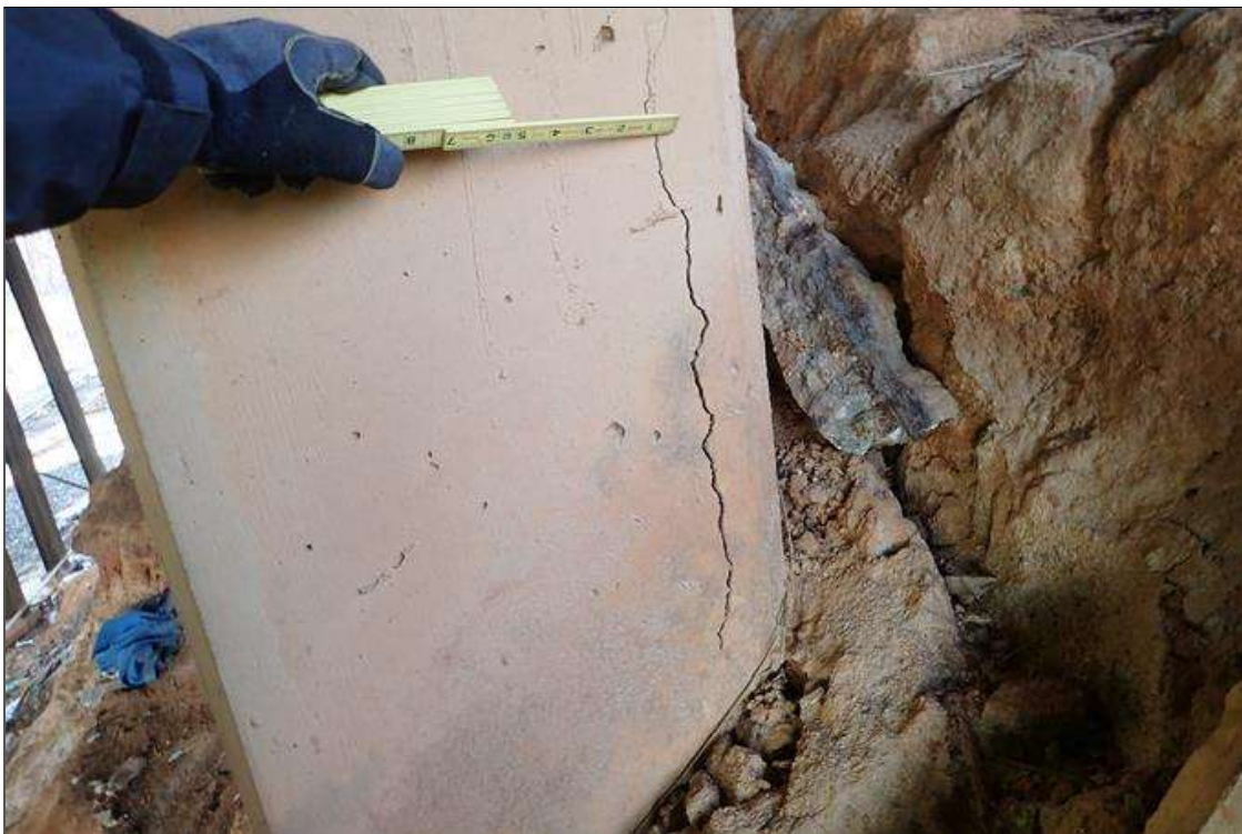
Bent 4 Pile 15: vertical crack (1/8" x 2')
