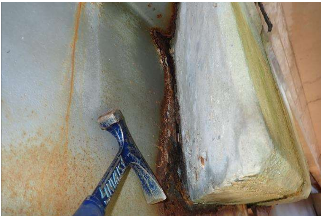
Span 1 Beam 11: (PAR) at bent 1, corrosion with section loss: bottom flange, (0.6" average remaining x 3'); web at end diaphragm, (1/8" remaining x 3" wide x 19")
