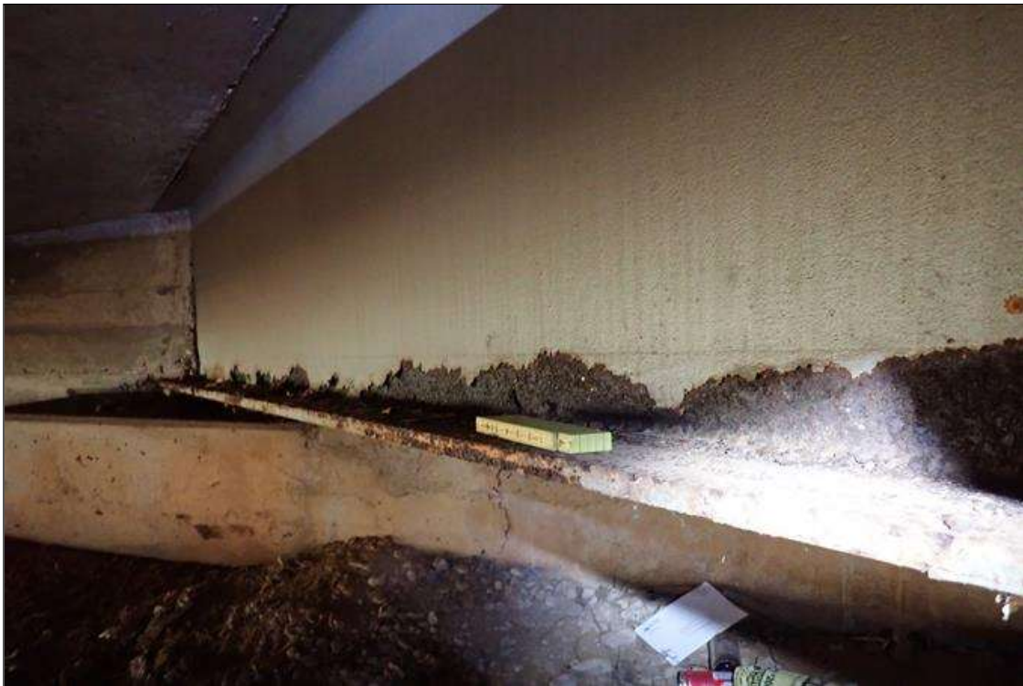
Span 1 Beam 7: at end bent 1, bottom of web, corrosion with section loss (7/16" remaining x 4" x 10')
