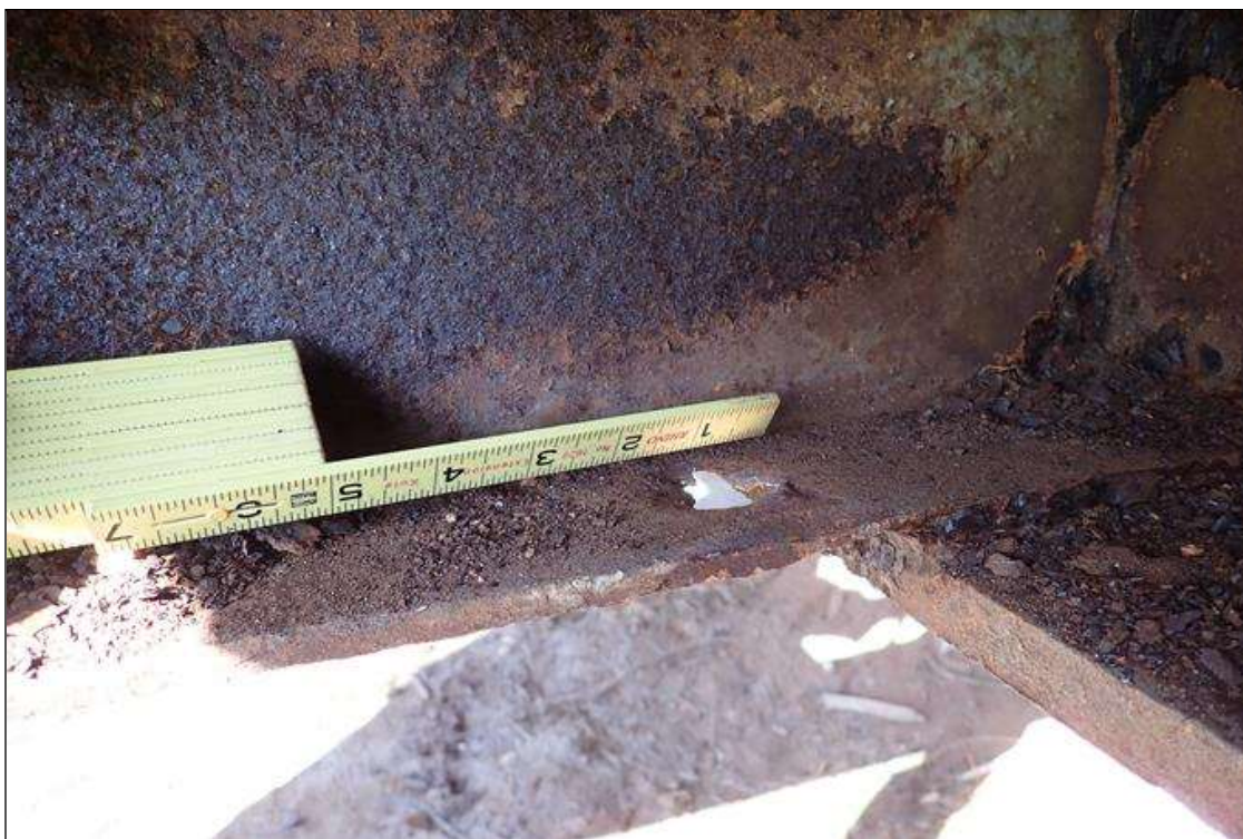
(PAR) span 1 utility, right overhang, 6' from bent 1, section loss on clamp rods (5/8" remaining); and bottom flange of bracket at beam, corrosion hole (1.5" diameter)
