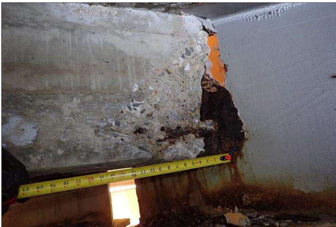
Span 1 Deck: bent 1 end diaphragm, bay 7 at beam 8, spall (16" x 18" x 2") with exposed rusted rebar
