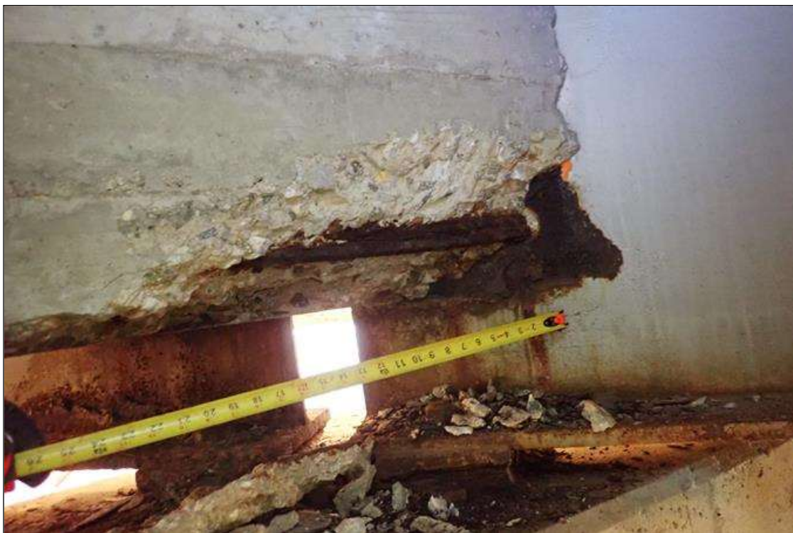
Span 1 Deck: bent 1 end diaphragm, bay 8 at beam 9, spall (30" x 8" x 4") with exposed rusted rebar, similar at beam 8
