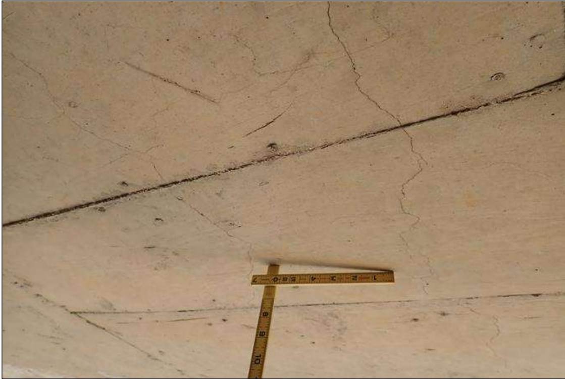
Span 2 Deck: underside at bent 4, bays 9 and 10, multiple transverse cracks (hairline up 1/32" x 7')
