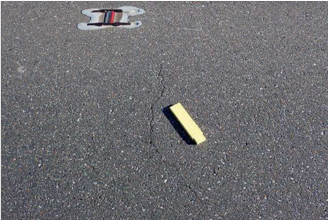
Span 1 Wearing Surface: at random, transverse cracks (up to 1/8" x 3')
