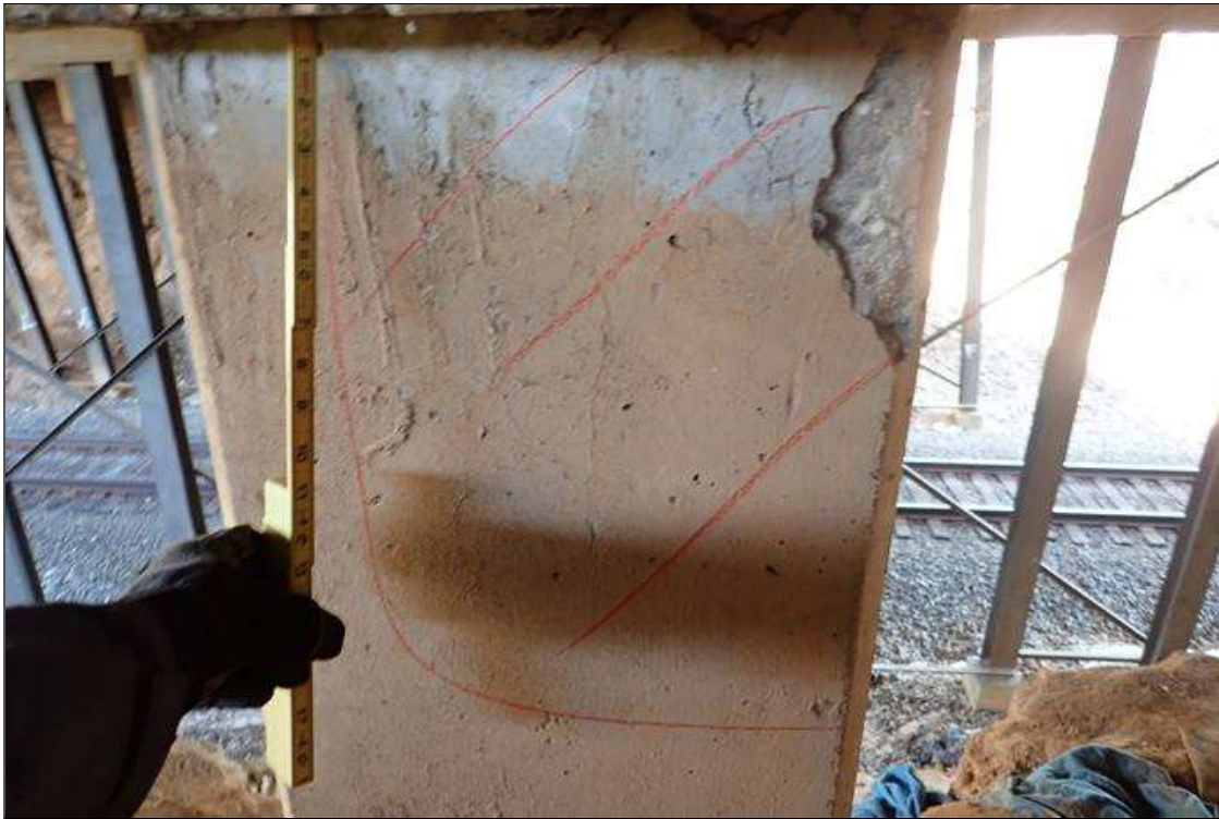
Bent 4 Pile 14: span 5 face, at top, delamination/spall (15" x 18" x 1/2")
