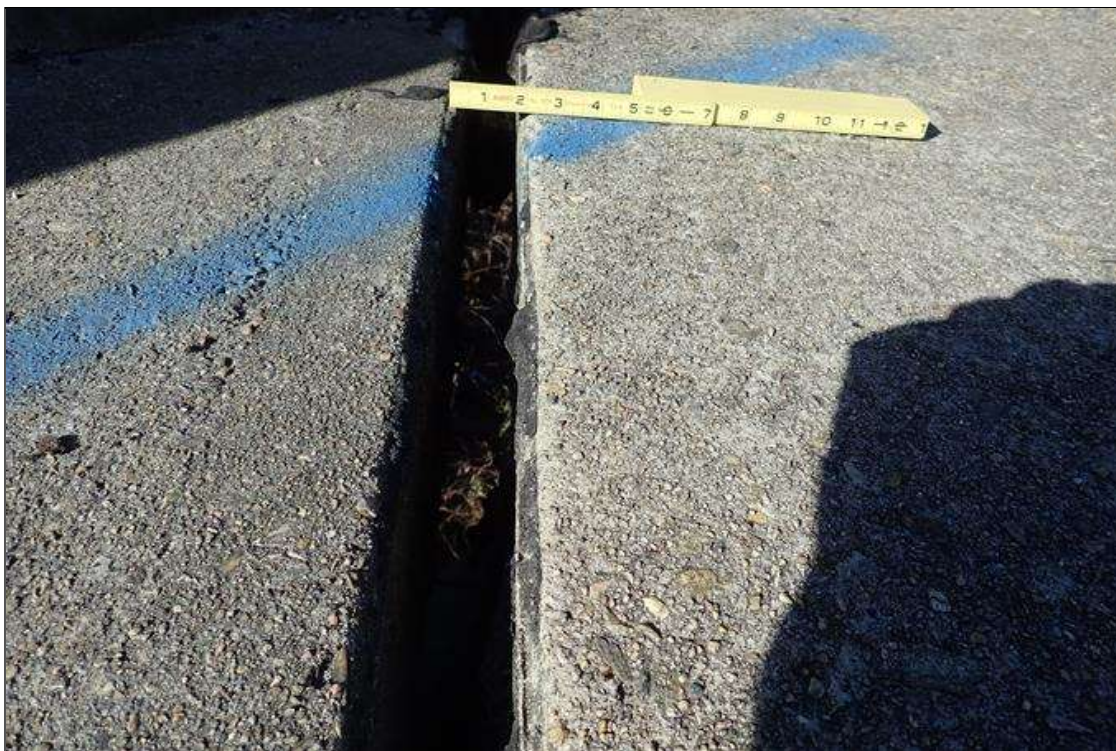
Bent 4 Joint : at right sidewalk, joint material missing
