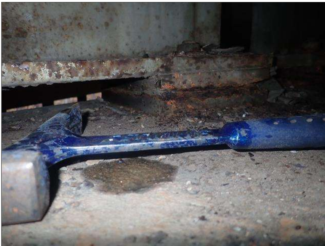
Span 4 Beam 8 Far Bearing 8: (PAR) bearing frozen with pack rust
