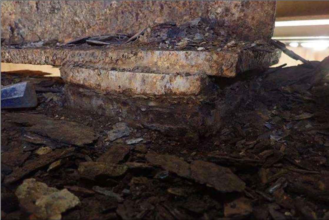
Span 4 Beam 7 Far Bearing 7: (PAR) bearing frozen with pack rust
