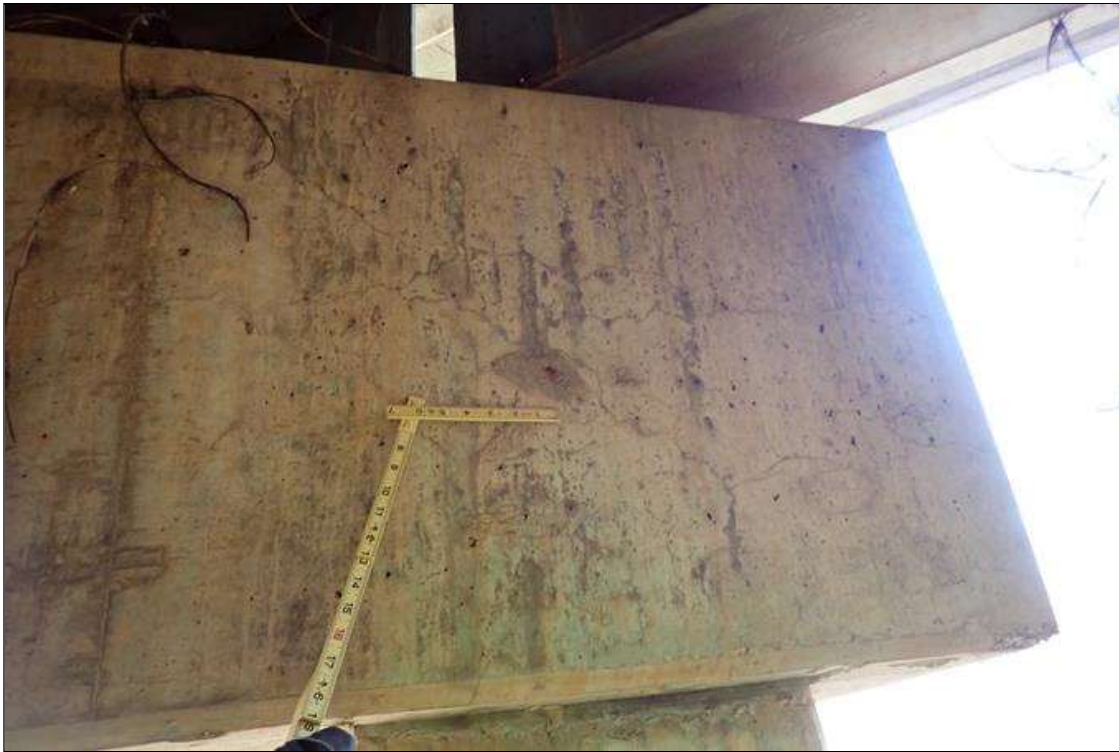
Bent 4 Cap 1: left end, map cracks (hairline x 2' x full height)
