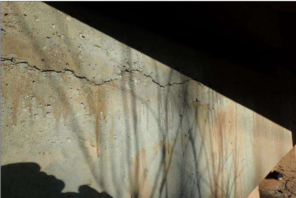
Bent 1 Cap 1: span 2 face, below beams 7 - 11, longitudinal crack (1/8" x 48') with areas of delaminations/spalls (up to 2' high x 1/2" deep), with some rust stains
