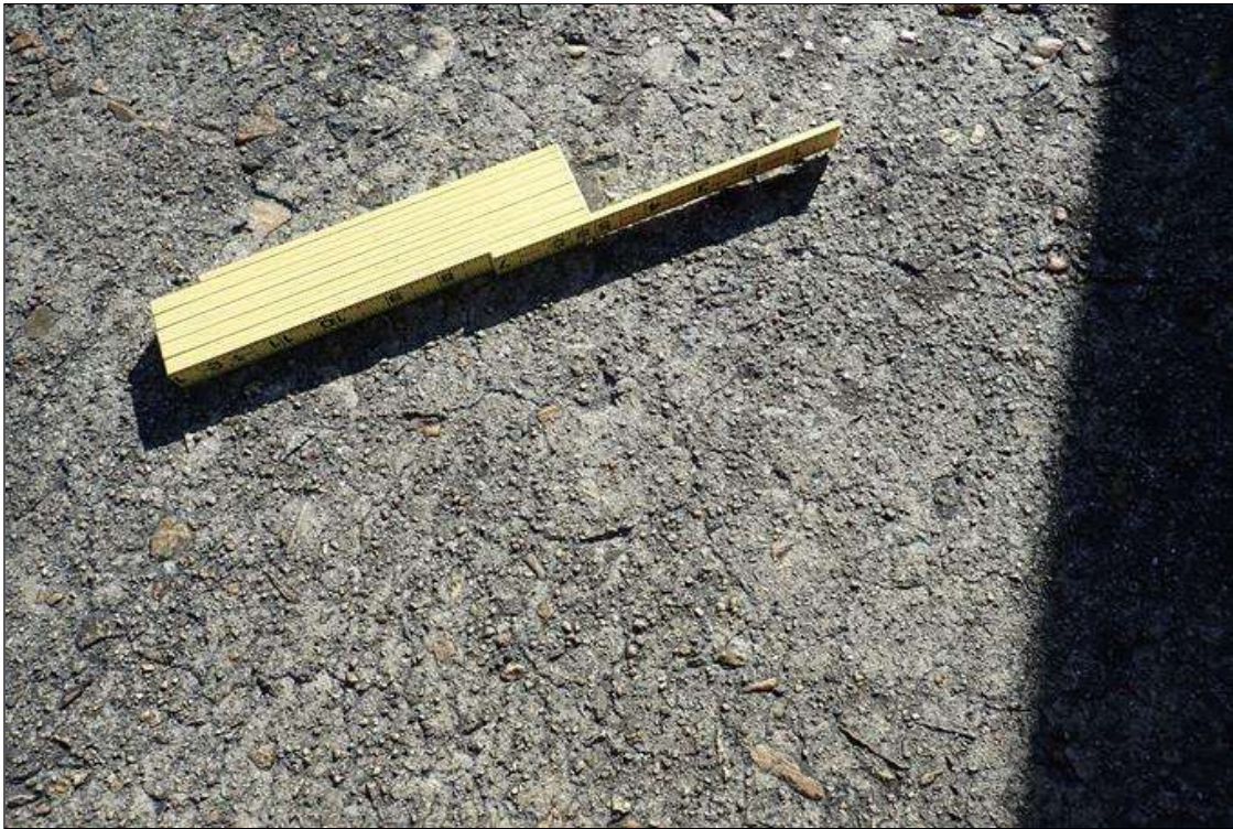
Span 4 Right Bridge Rail: throughout sidewalk and end post, map cracks (up to 1/32")
