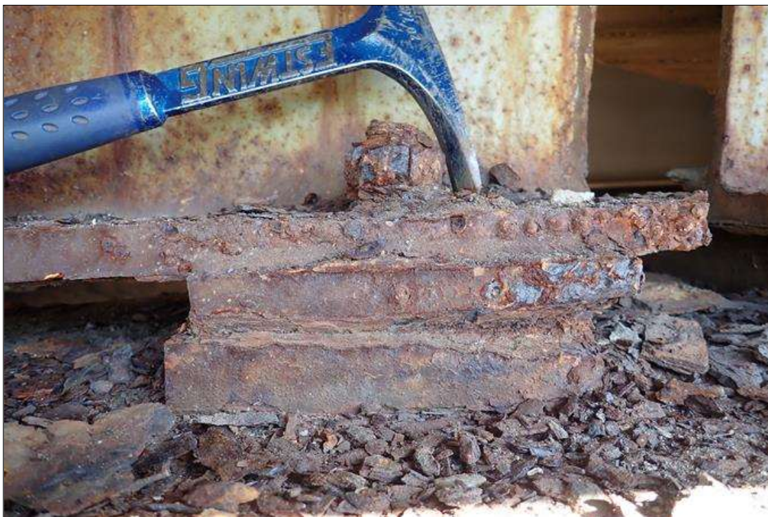
Span 1 Beam 11 Far Bearing 11: (PAR) bearing frozen with pack rust
