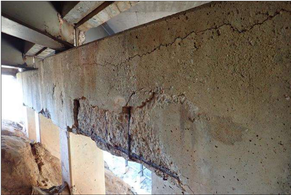
Bent 4 Cap 1: (PAR) span 5 face, from beam 8 to 11, longitudinal cracks (1/8" x 30') at top and bottom corners with delamination (up to full height x 30') and spalls (19' x up to 20" x 2") with exposed rusted rebar; cracks and delamination similar on span 4 face
