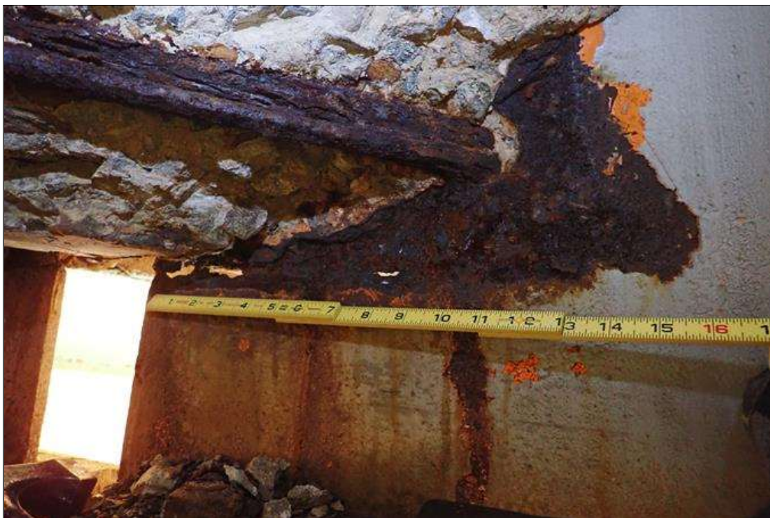
Span 1 Beam 9: (PAR) at bent 1 end diaphragm, corrosion with section loss: web, (1/8" remaining x 16" x 8") with corrosion hole (9" x 1/2")
