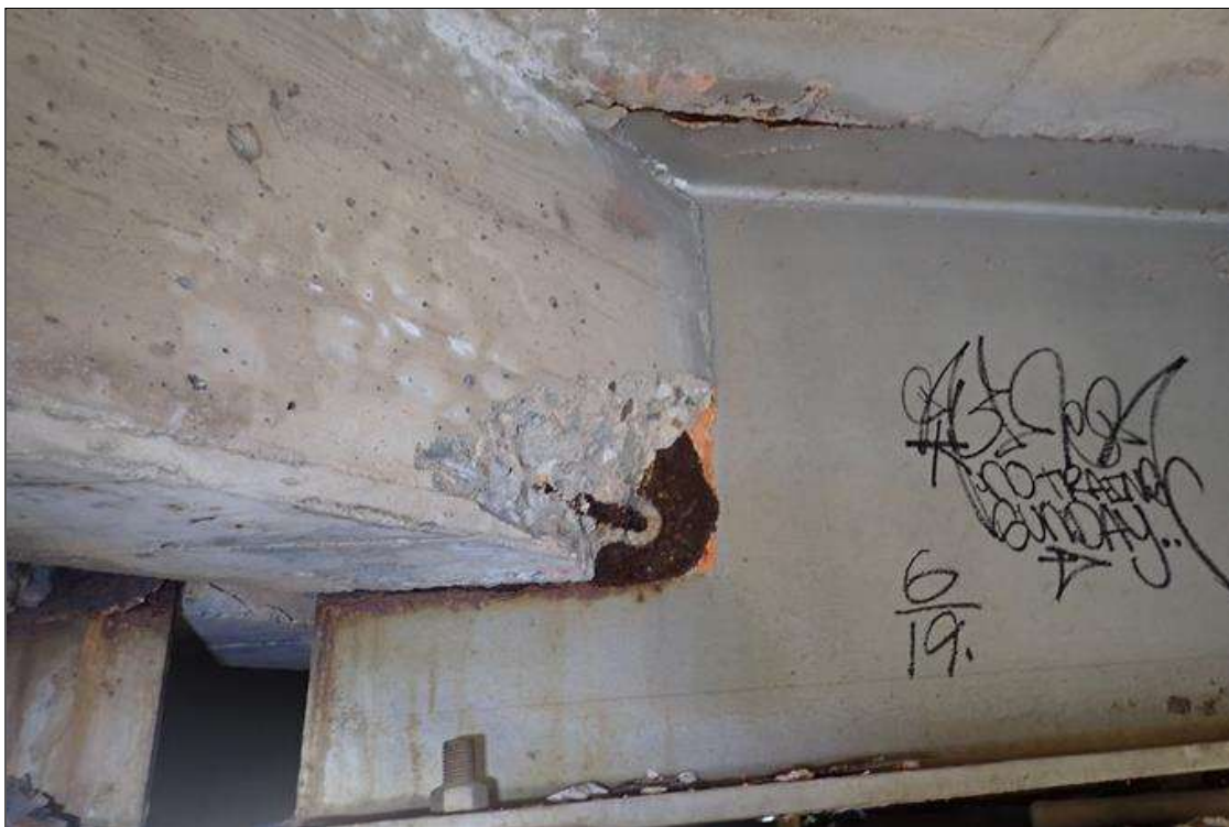
Span 2 Deck: bent 1 end diaphragm, bay 10, at beam 10, spall (1' x 8" x 2") with exposed rusted rebar
