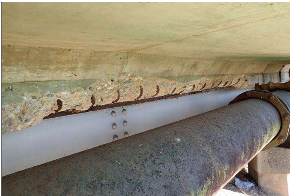
Span 1 Deck: (PAR) right side of beam 11 haunch, at bent 2, spall (14' x 6" x 5") with exposed rusted rebar
