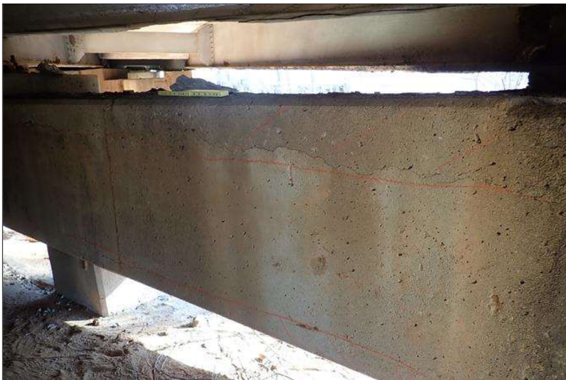
Bent 1 Cap 1: span 1 face, top corner, longitudinal crack (1/16" x 9') with delamination/spall (6" x 1"), similar bottom corner
