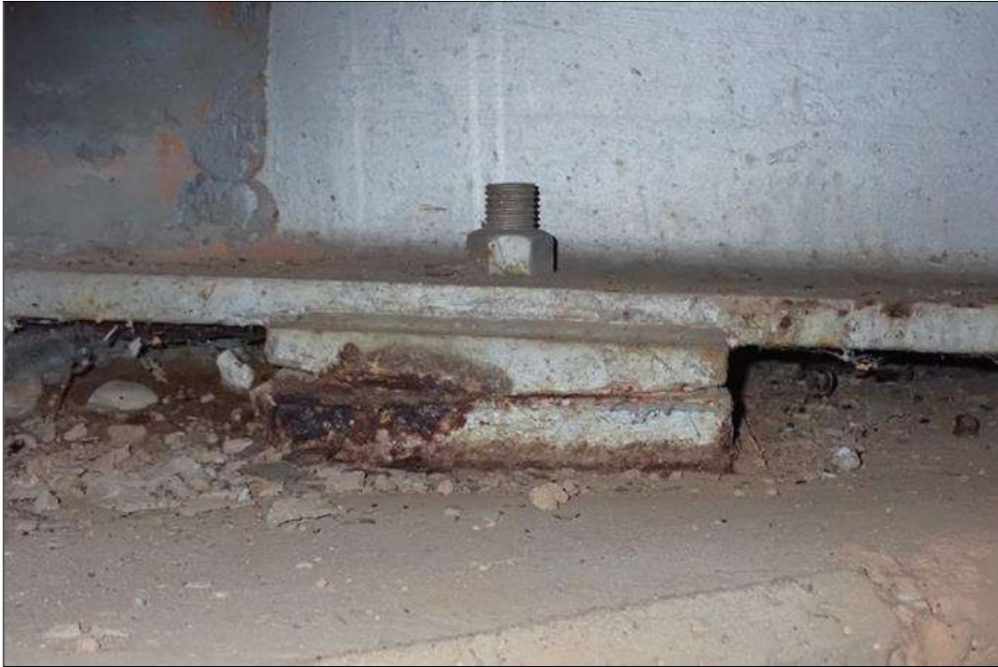
Span 5 Beam 8 Far Bearing 8: rust scale
