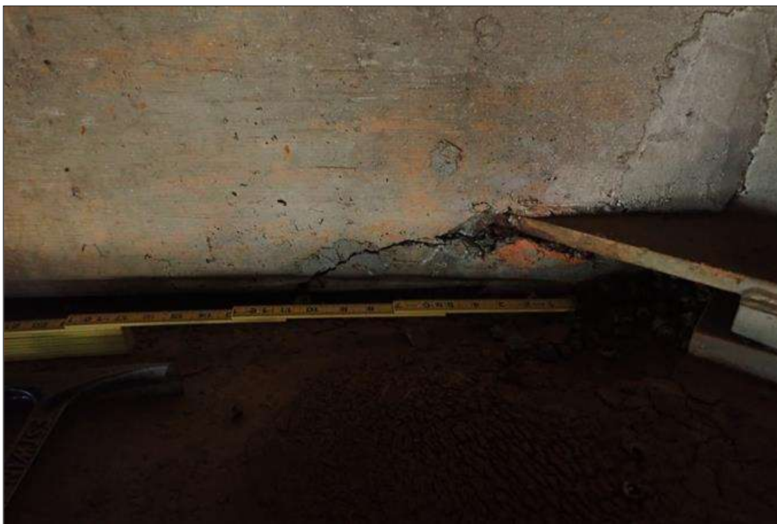
End Bent 2 Abutment/Backwall : bay 6, at beam 7, bottom flange, spall (12" x 3" x 1")
