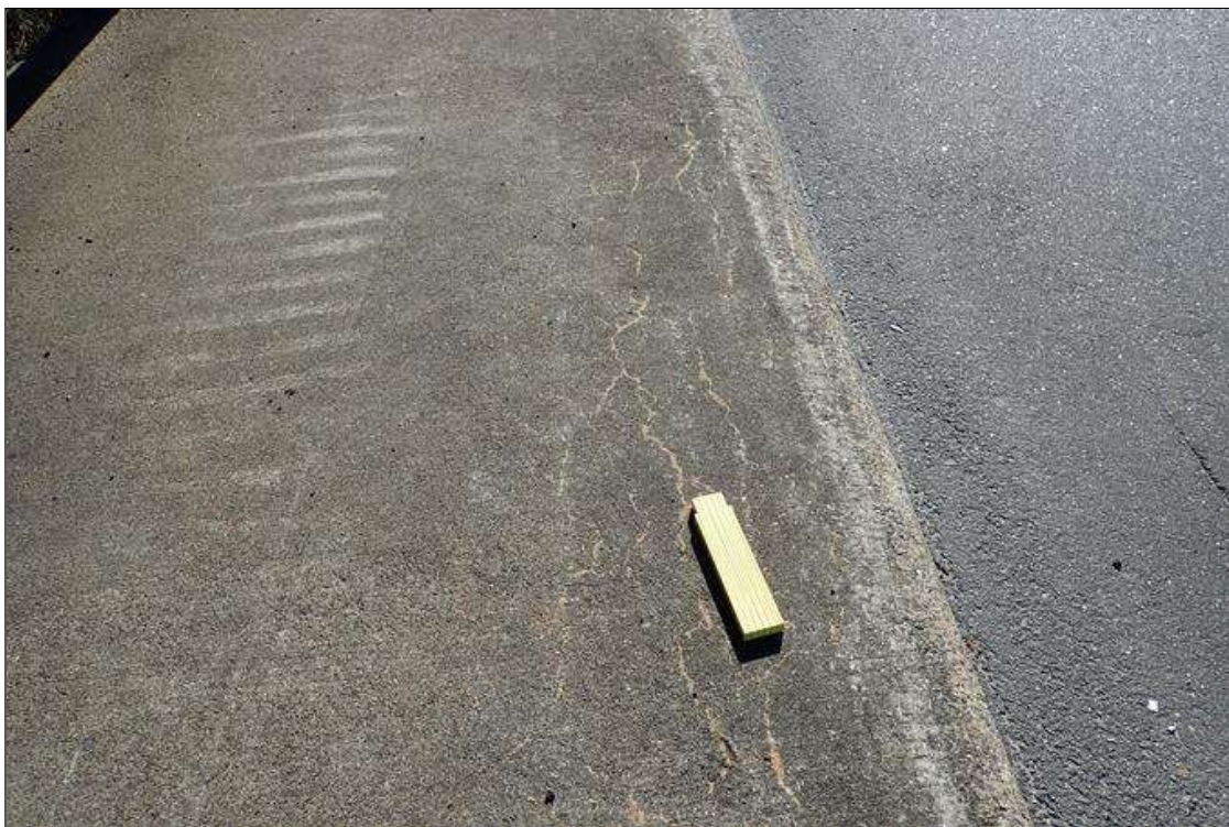
Span 1 Left Bridge Rail: along edge of sidewalk, map cracks (hairline x 1' x full length)
