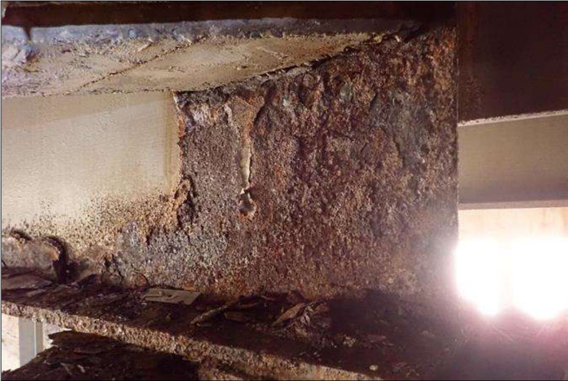
Span 4 Beam 7: (PAR) at bent 4, corrosion with section loss: web, at bearing, (3/8" remaining x 16" x 12"); bottom of web, (1/4" remaining x 2" x approximately 15'); bottom flange, (0.7" average remaining x 16")
