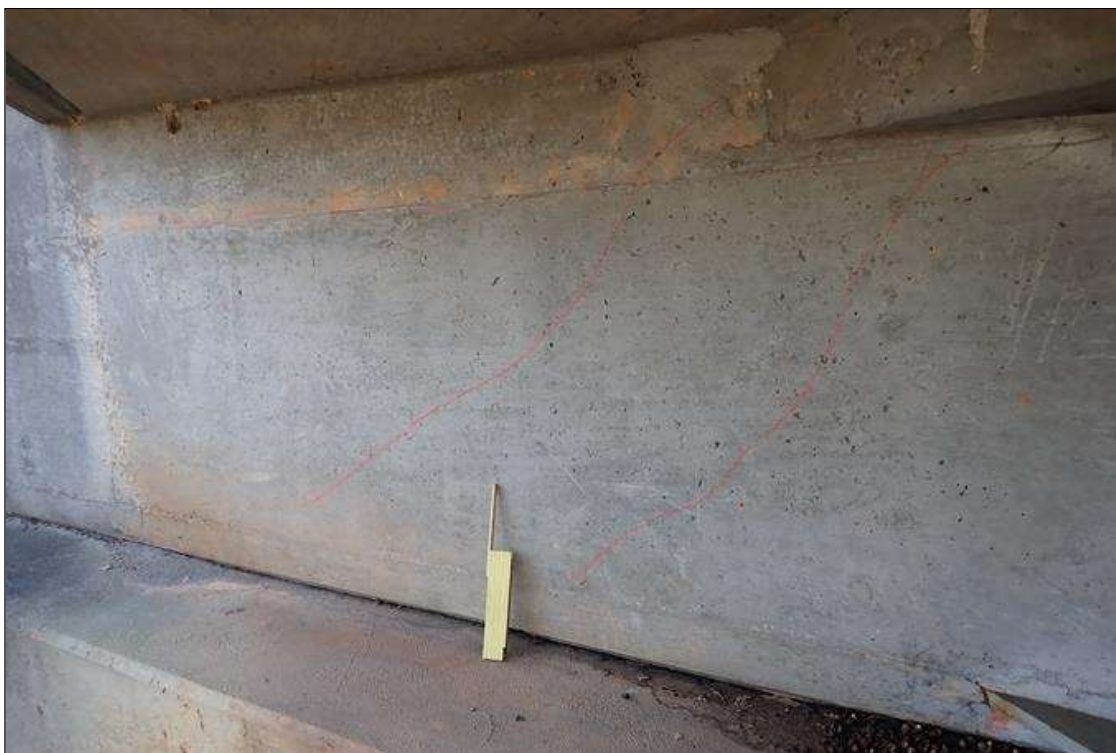
End Bent 2 Abutment/Backwall : left end, (3) diagonal cracks (1/32" x 5') with map cracks (hairline)
