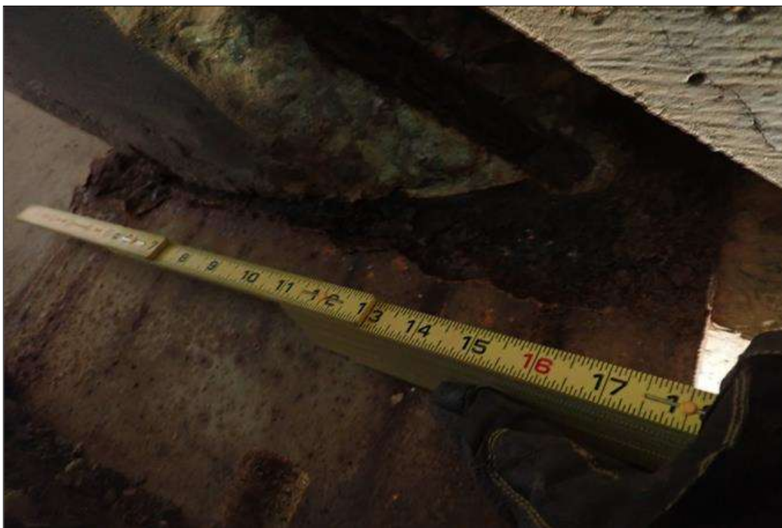
Span 2 Beam 10: (PAR) at bent 1, corrosion with section loss: web at end diaphragm, (1/16" remaining x 18" x 7")
