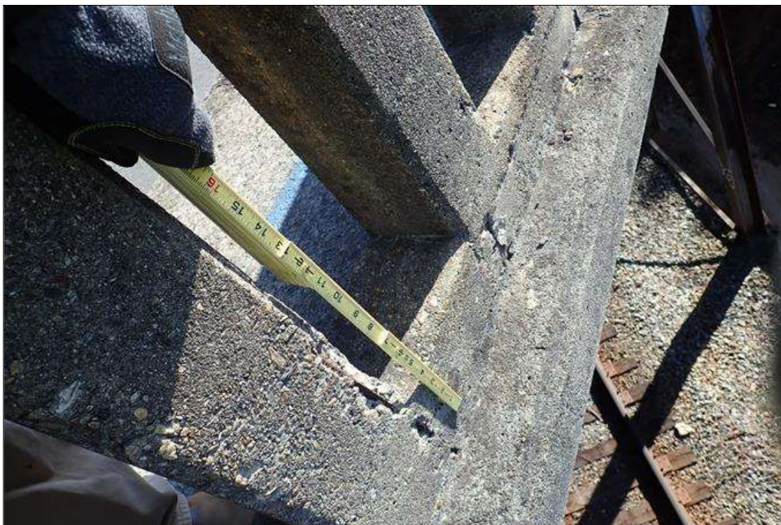
Span 3 Right Bridge Rail: rail posts at random, (10) spalls (up to 16" x 2" x 1/2") with exposed rusted rebar
