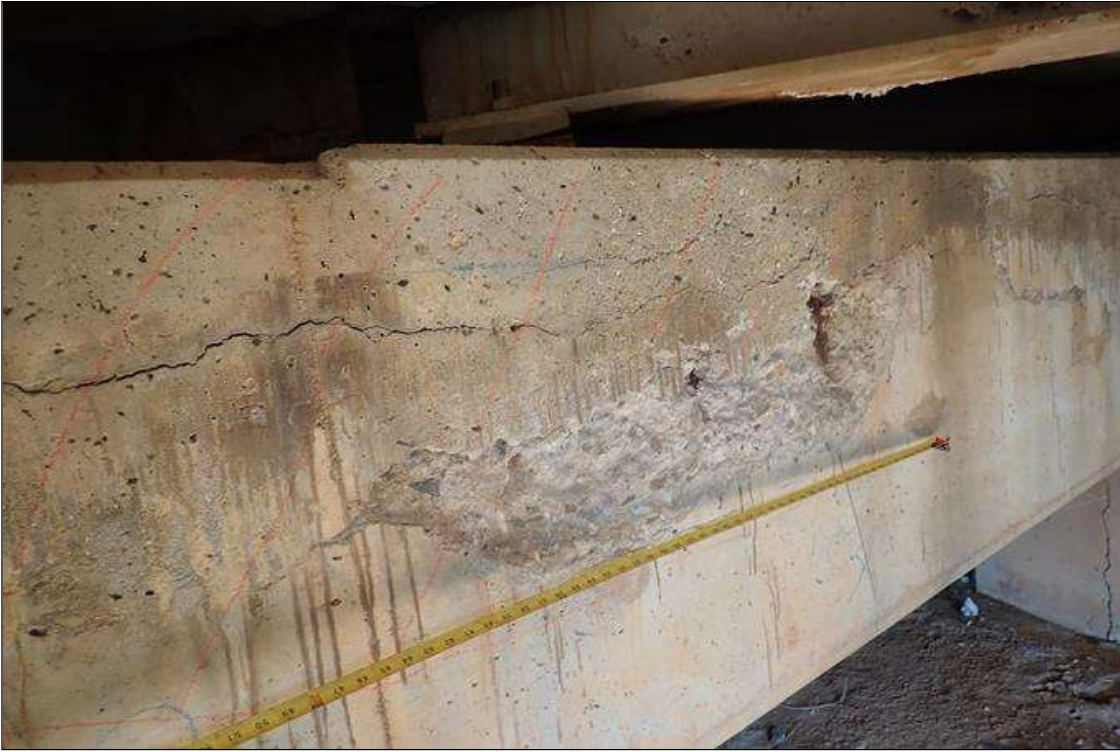
Bent 1 Cap 1: span 2 face, below beam 9, spall/delamination (5' x 2' x 1.5") with exposed rusted rebar
