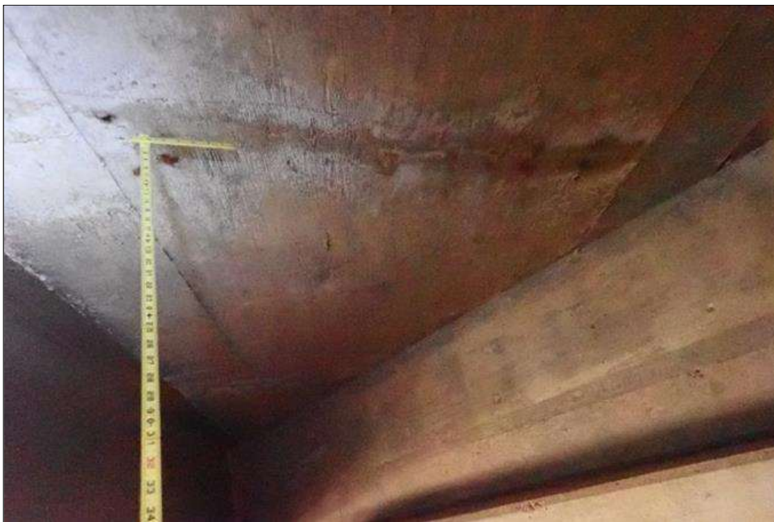
Span 1 Deck: underside of deck at end bent 1, bay 5, diagonal crack (hairline x 6') with efflorescence, similar bays 2 and 4
