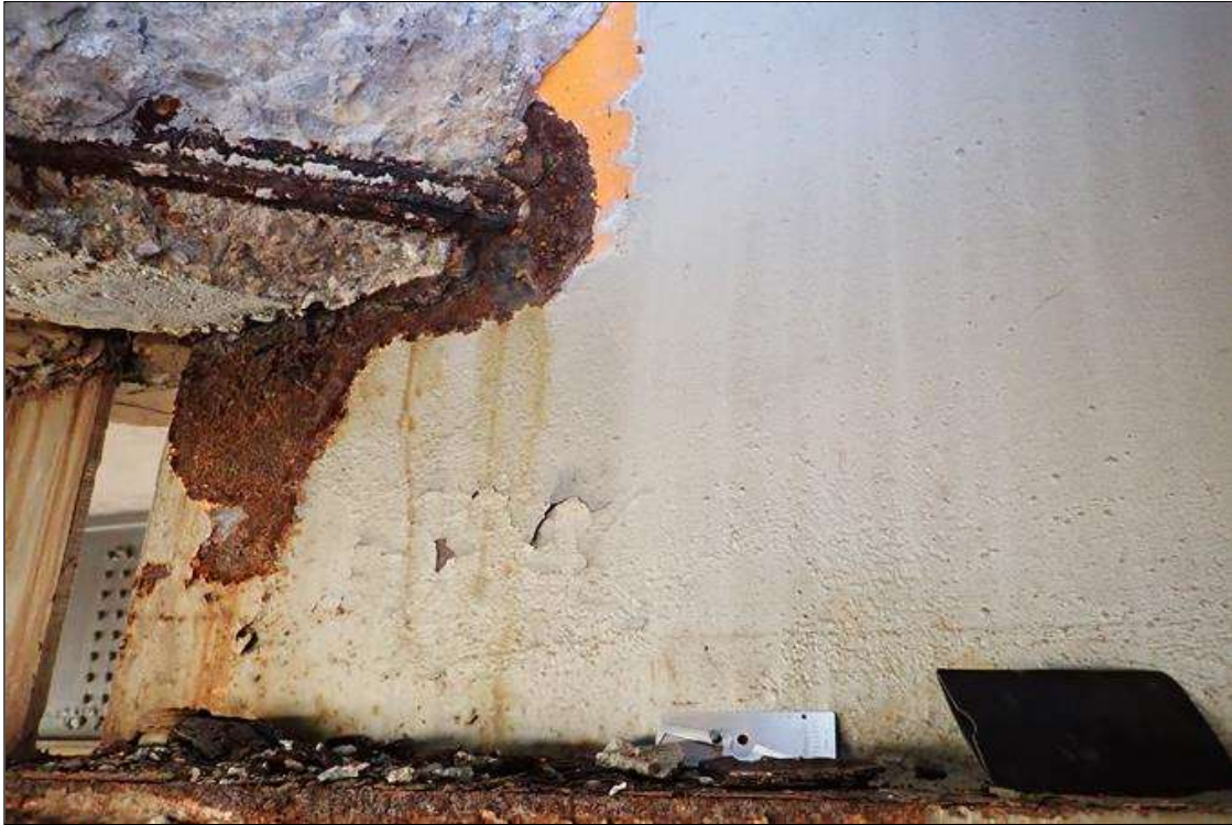
Span 5 Beam 9: (PAR) at bent 4, corrosion with section loss: web at end diaphragm, (1/4" remaining x 14" x 5"); bottom flange, pitting (up to 1/16" x 1.5')
