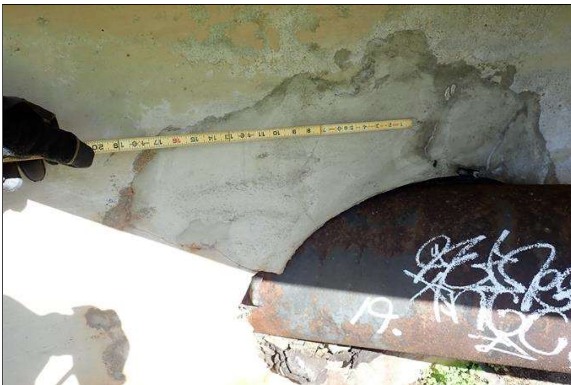
End Bent 1 Abutment/Backwall : right overhang at utility penetration, map cracks (hairline) with efflorescence
