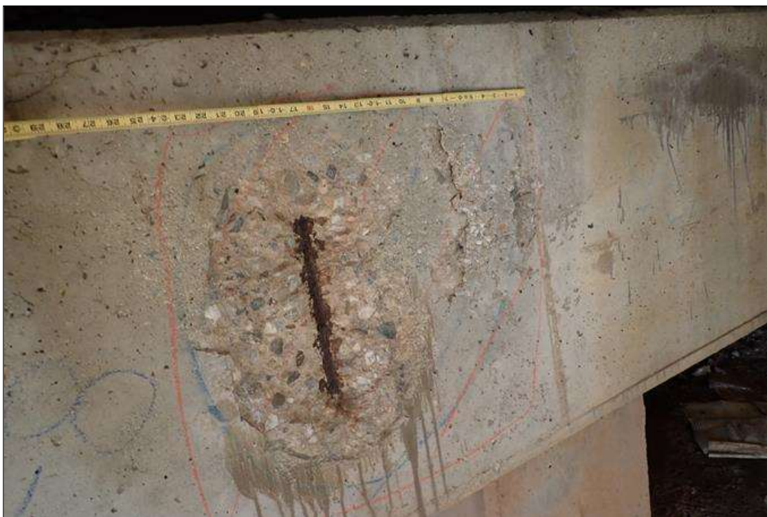
Bent 1 Cap 1: span 2 face, below beam 8, spall/delamination (2' x 2' x 1") with exposed rusted rebar
