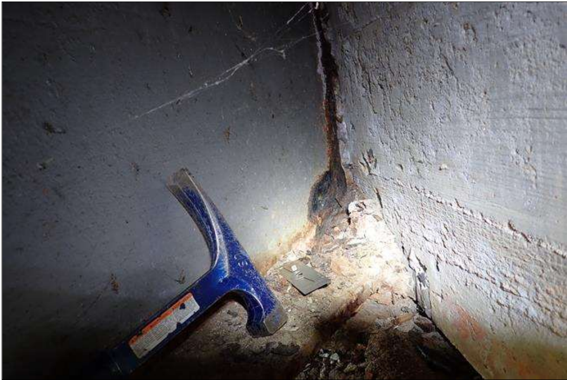
Span 1 Beam 11: (PAR) at end bent 1, bottom of web, left face, corrosion with section loss (1/4" remaining x 8" x 6")
