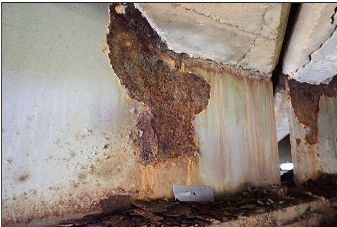
Span 4 Beam 9: (PAR) at bent 4, corrosion with section loss: web at end diaphragm, (1/4" remaining x 1.5' x up to 12")
