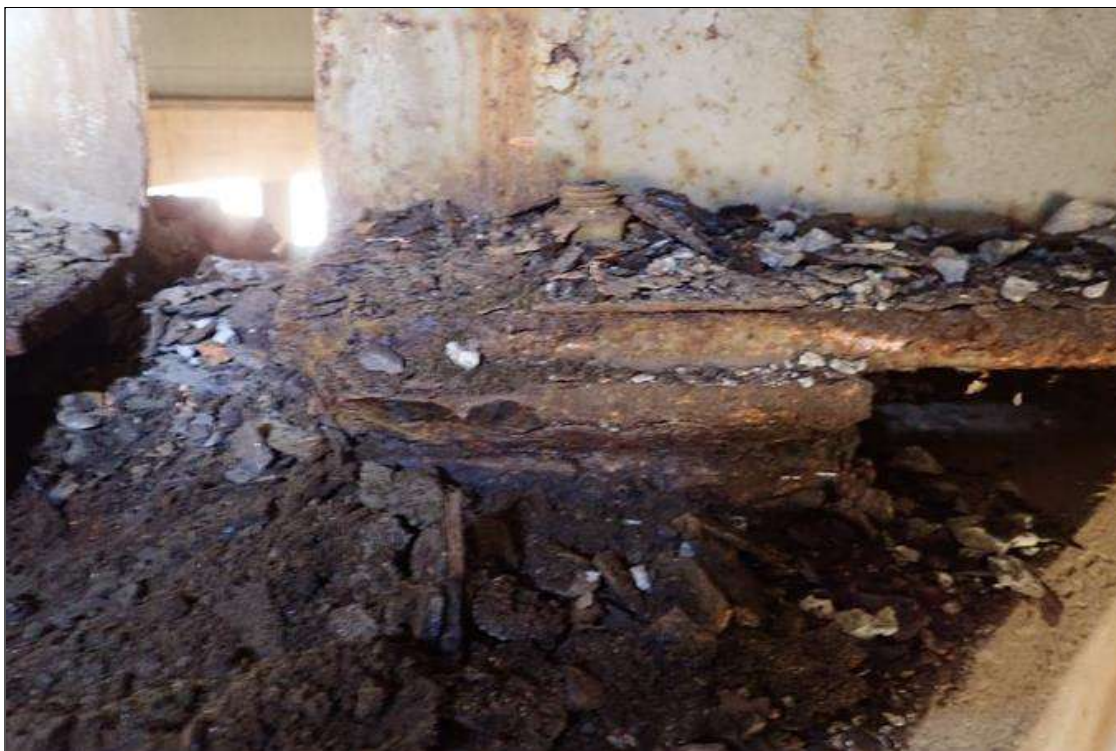
Span 5 Beam 9 Near Bearing 9: (PAR) bearing frozen with pack rust
