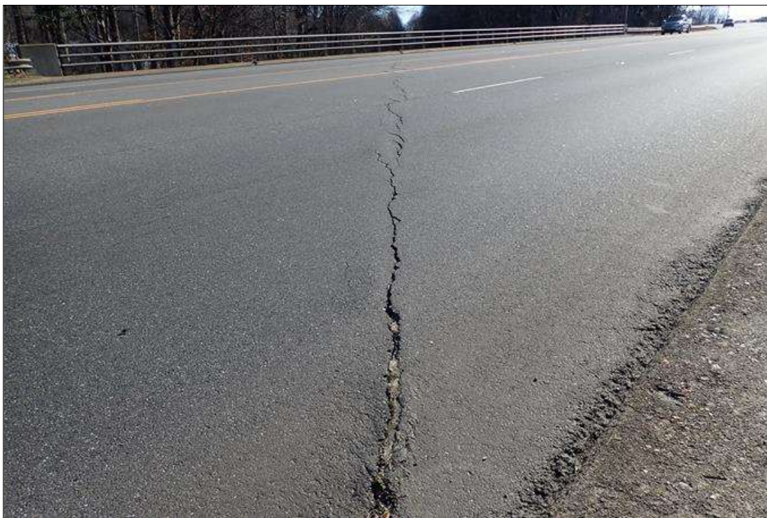
Span 2 Wearing Surface: UP TO 0.5" TRANSVERSE CRACKS OVER BENT 2
