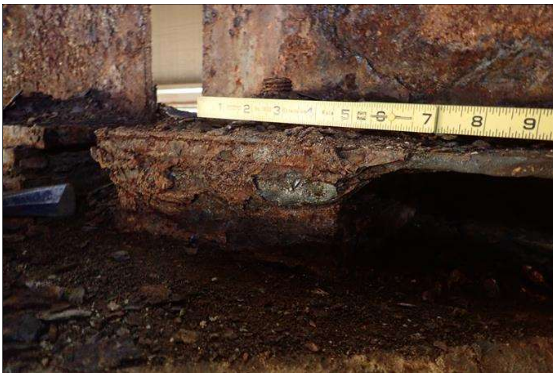
Span 5 Beam 7 Near Bearing 7: (PAR) bearing frozen with pack rust and 1/8" section loss at edge of plate
