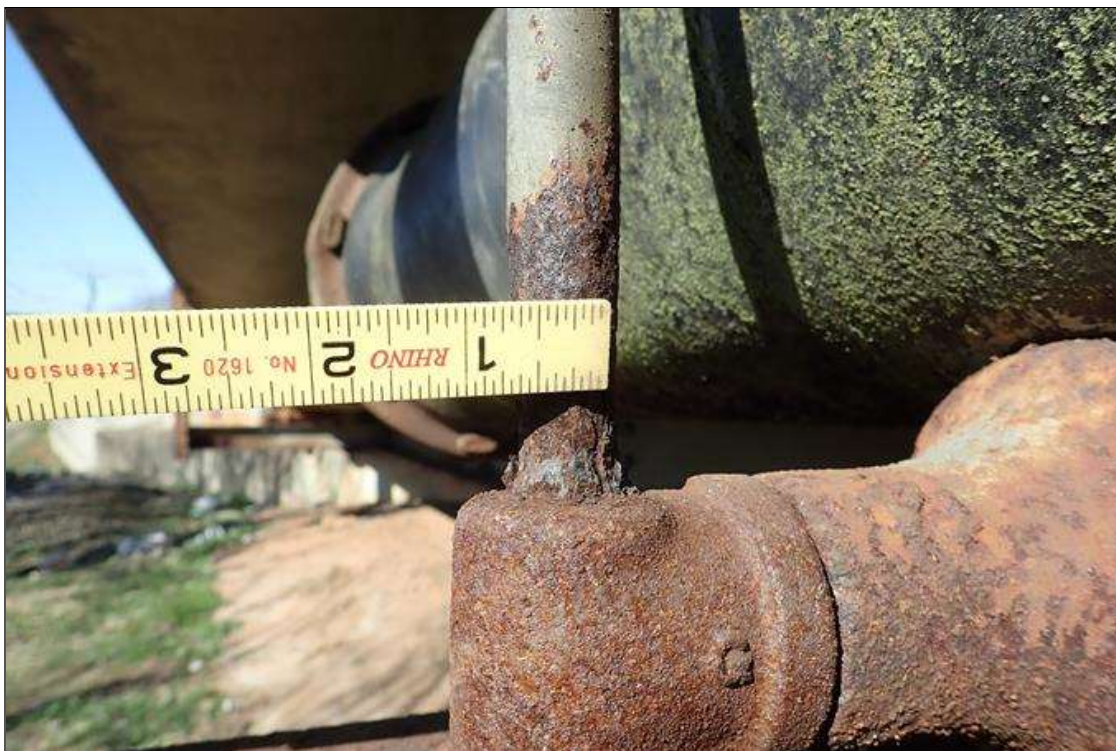
(PAR) span 1 utility, right overhang, 6' from bent 1, section loss on clamp rods (5/8" remaining); and bottom flange of bracket at beam, corrosion hole (1.5" diameter)
