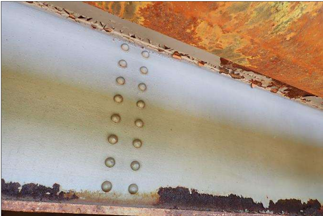
Span 1 Beam 11: both flanges, below deck haunch spall, rust scale with pitting (up to 1/16")
