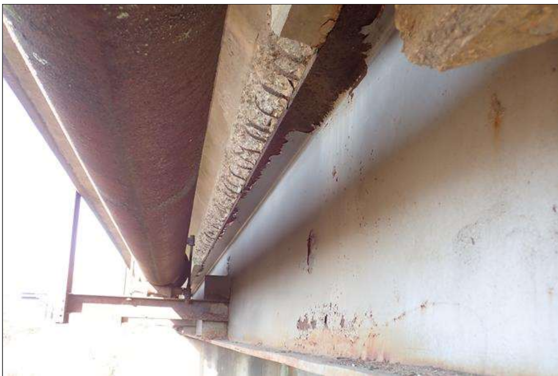
Span 4 Deck: (PAR) at bent 4, right side of beam 11 haunch, spall (25' x 5" x 5") with exposed rusted rebar
