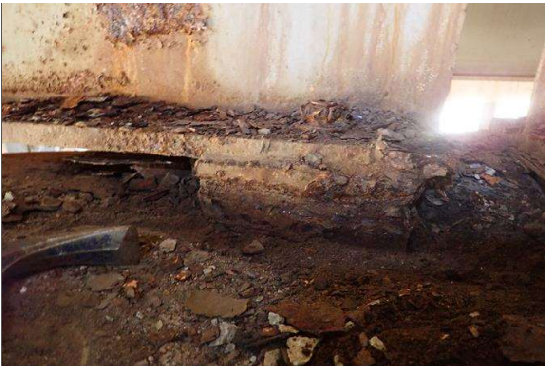
Span 4 Beam 9 Far Bearing 9: (PAR) bearing frozen with pack rust
