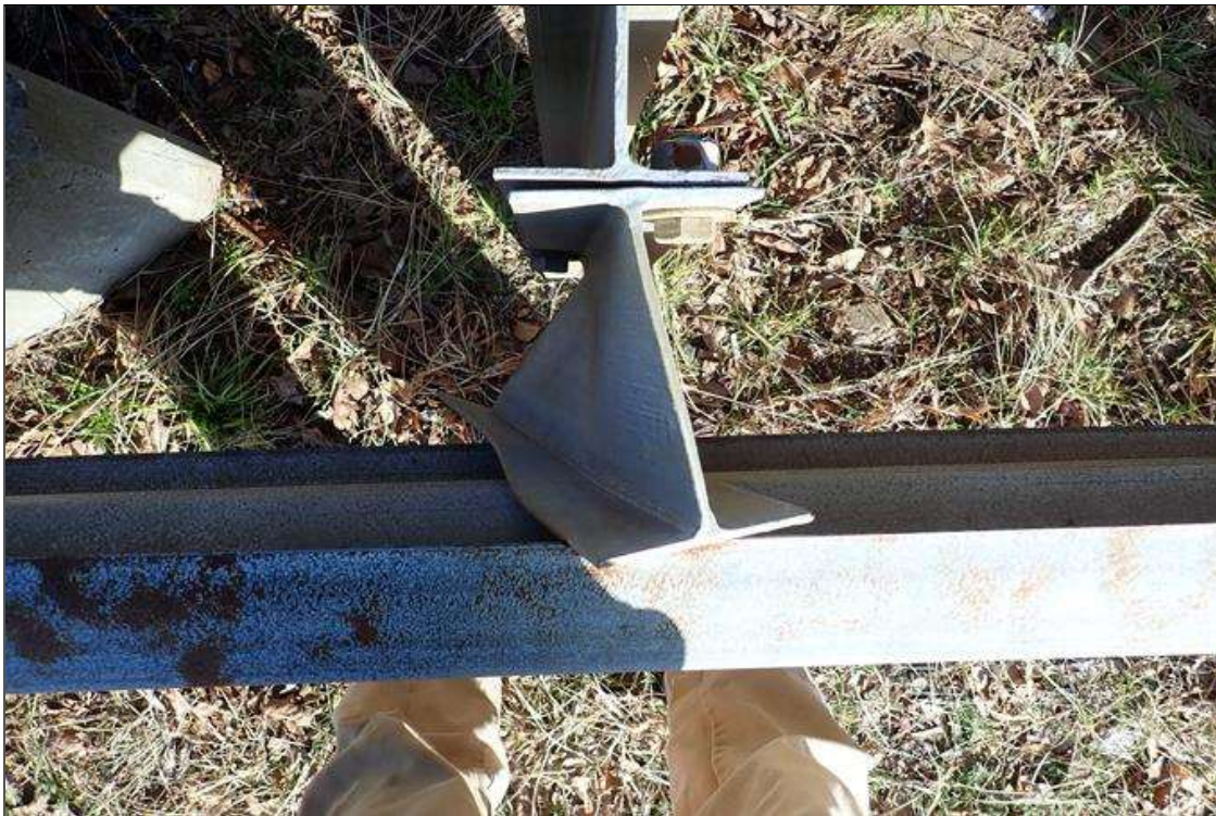
(PAR) northeast guardrail, near end bent 2, (2) spacer blocks twisted
