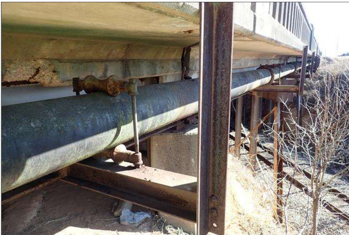
right overhang, throughout utility hangers, surface rust
