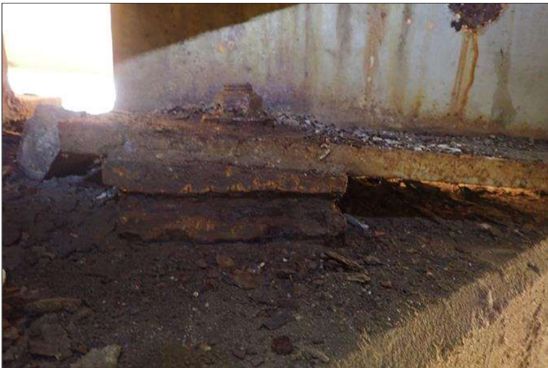
Span 1 Beam 10 Far Bearing 10: (PAR) bearing frozen with pack rust
