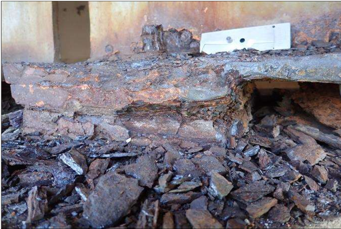
Span 5 Beam 11 Near Bearing 11: (PAR) bearing frozen with pack rust
