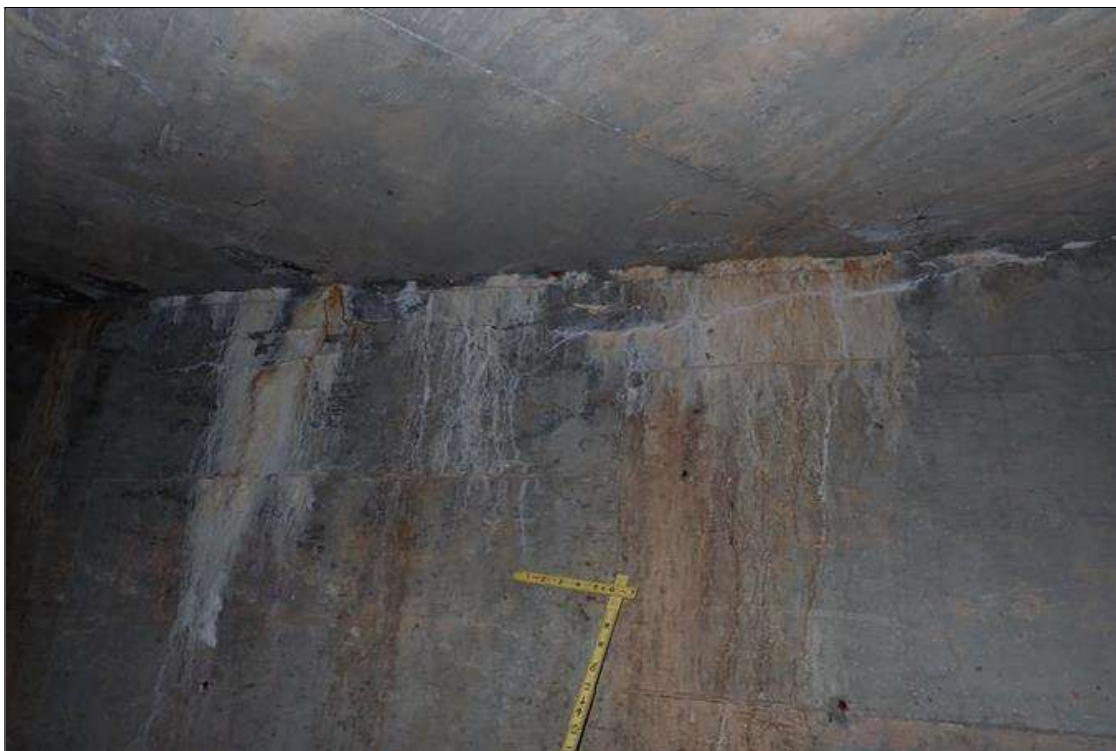
End Bent 2 Abutment/Backwall : bay 6, horizontal cracks (1/32" x 7') with efflorescence buildup
