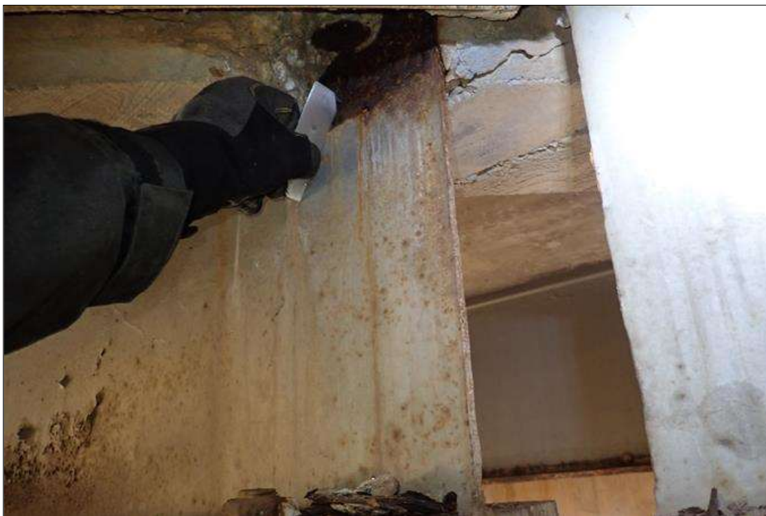
Span 4 Beam 8: (PAR) at bent 4, web at end diaphragm, (3/8" remaining x 6" x 4")
