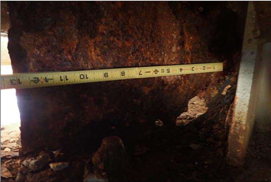
Span 1 Beam 7: (PAR) at bent 1, corrosion with section loss: web, corrosion hole at bearing (12" x 3"); bottom of web, (1/8" remaining x 4" x 11'), (5/16" remaining x 1" x next 6')
