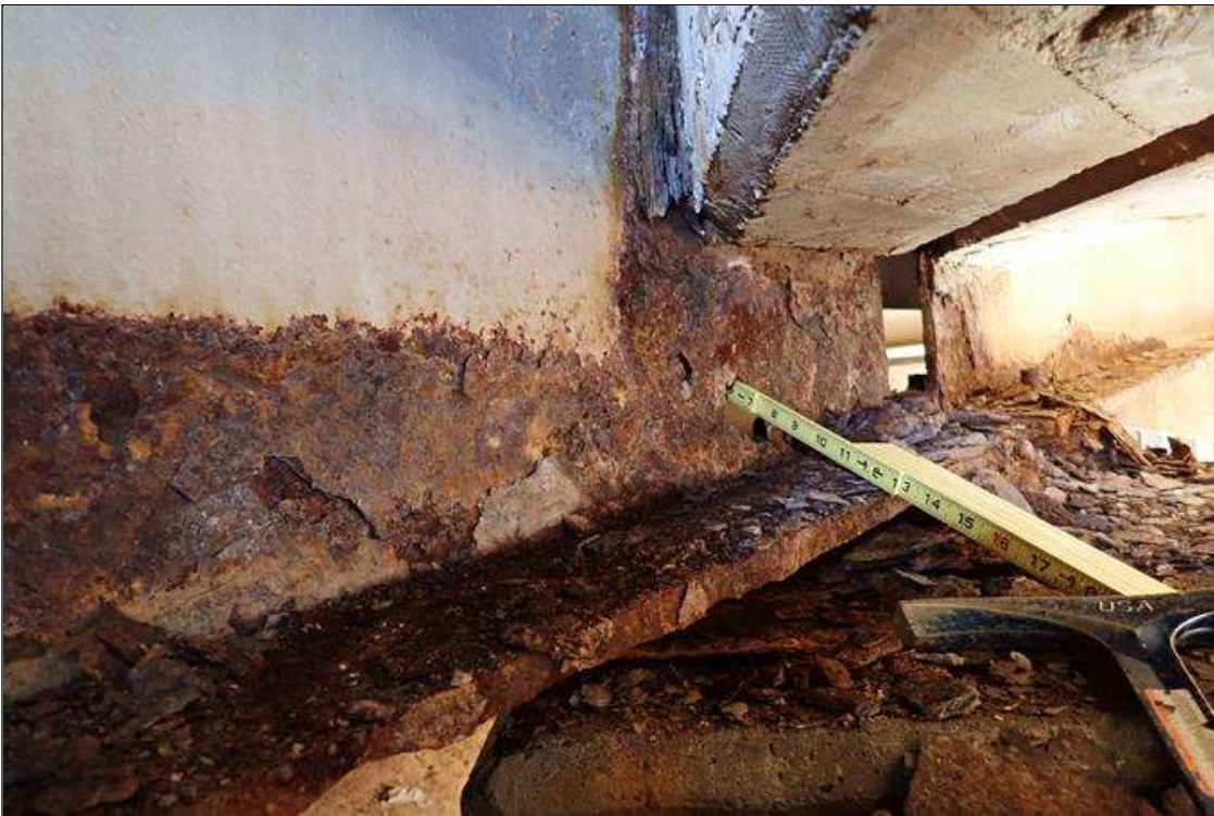
Span 1 Beam 7: (PAR) at bent 1, corrosion with section loss: web, corrosion hole at bearing (12" x 3"); bottom of web, (1/8" remaining x 4" x 11'), (5/16" remaining x 1" x next 6')
