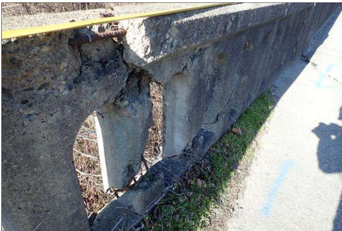
Span 5 Right Bridge Rail: (PAR) at bent 4, impact damage (14') with multiple broken posts and exposed rusted rebar
