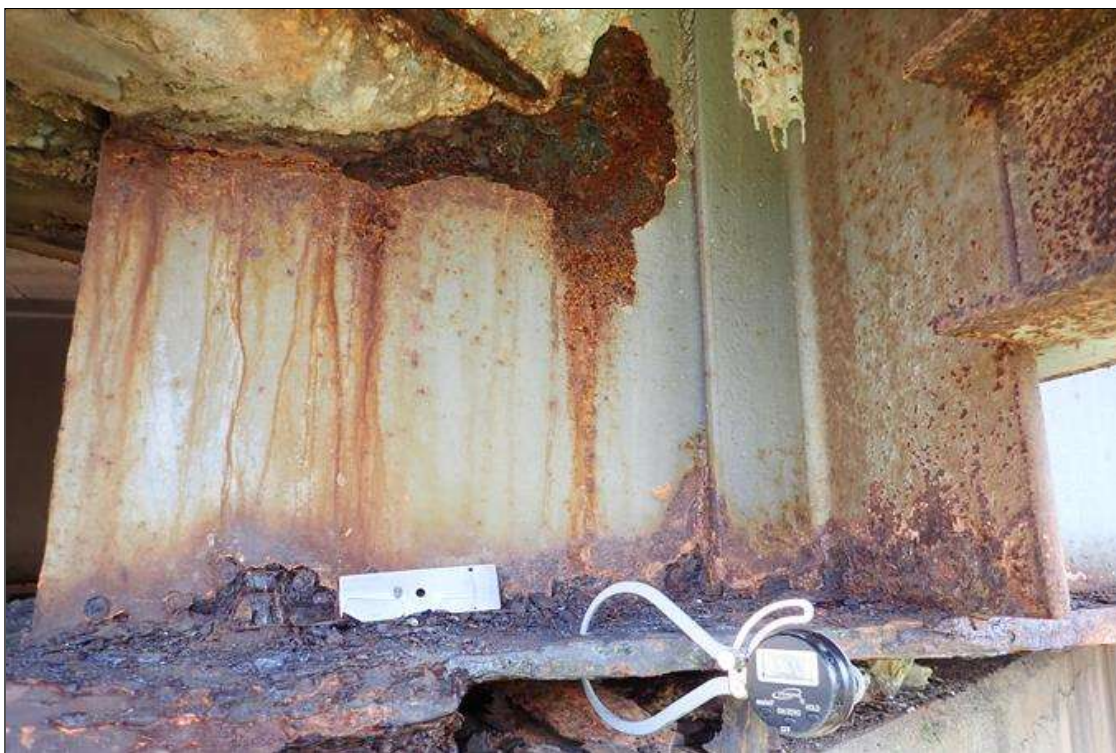
Span 5 Beam 11: (PAR) at bent 4, corrosion with section loss: bottom flange, (0.55" average remaining x 2'); web at end diaphragm, (1/16" remaining x 15" x 5")
