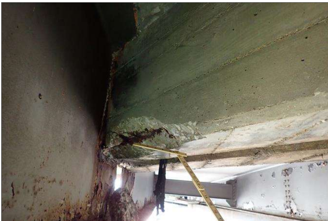
Span 5 Deck: bent 4 end diaphragm, bay 10, at beam 11, spall (18" x 3" x 4") with exposed rusted rebar
