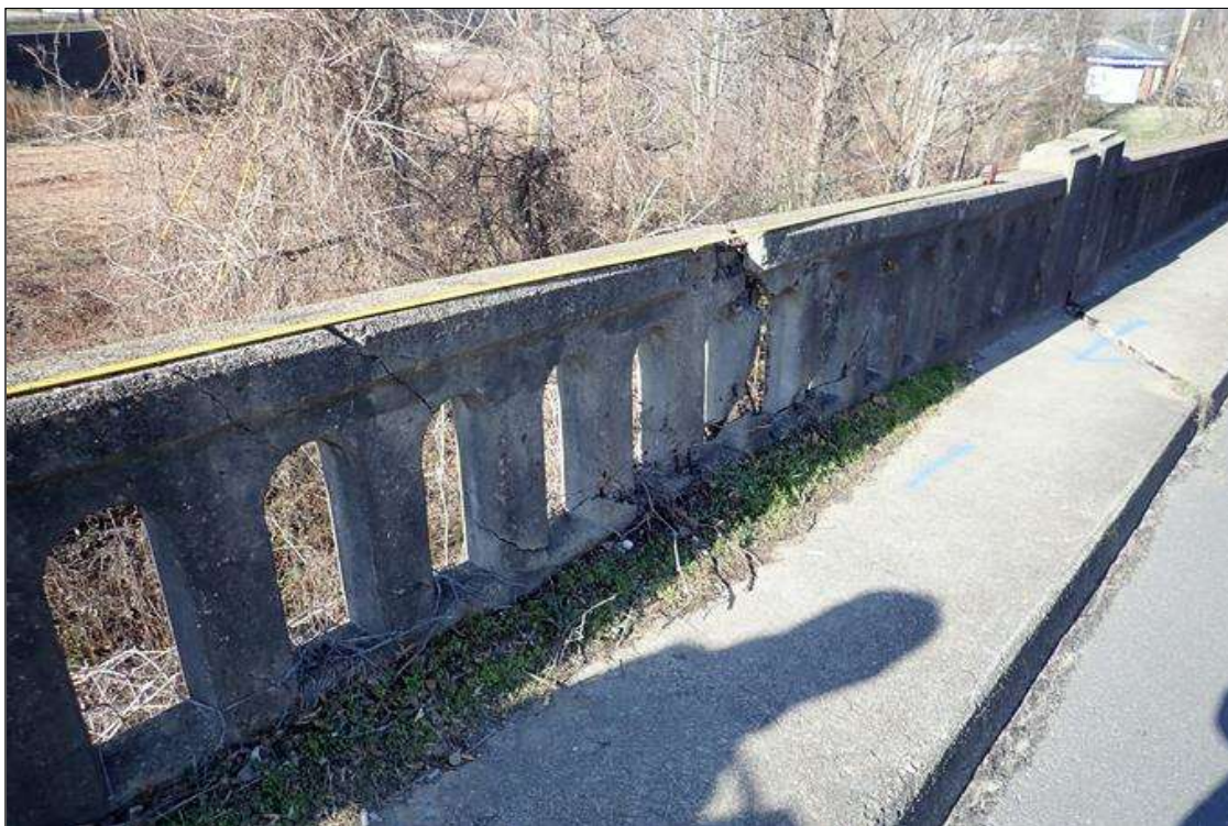
Span 5 Right Bridge Rail: (PAR) at bent 4, impact damage (14') with multiple broken posts and exposed rusted rebar
