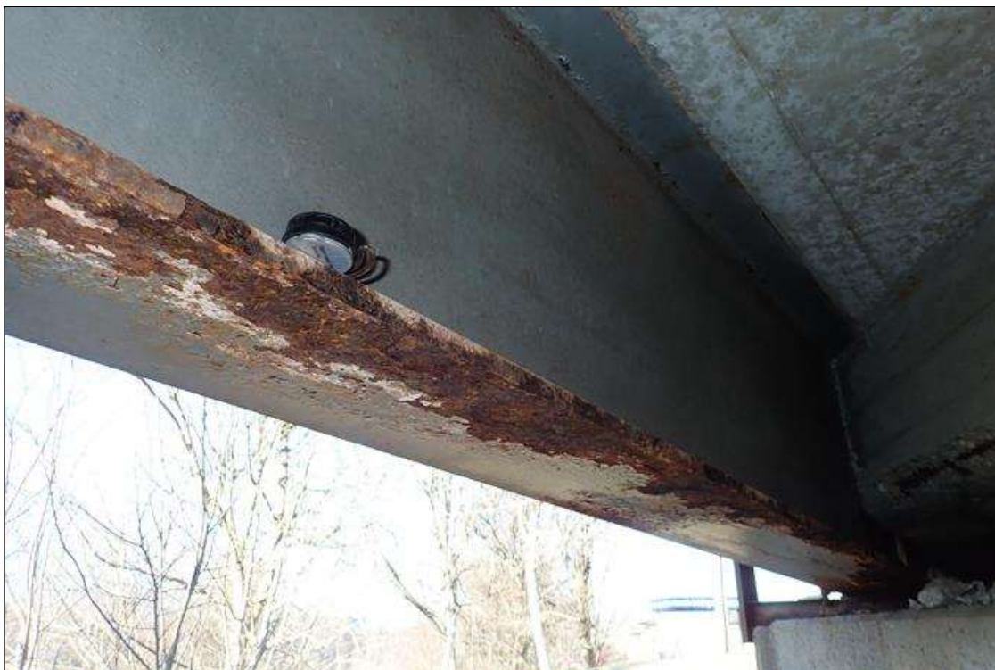
Span 2 Beam 11: at bent 1, bottom flange, corrosion with section loss (0.7" average remaining x 15')
