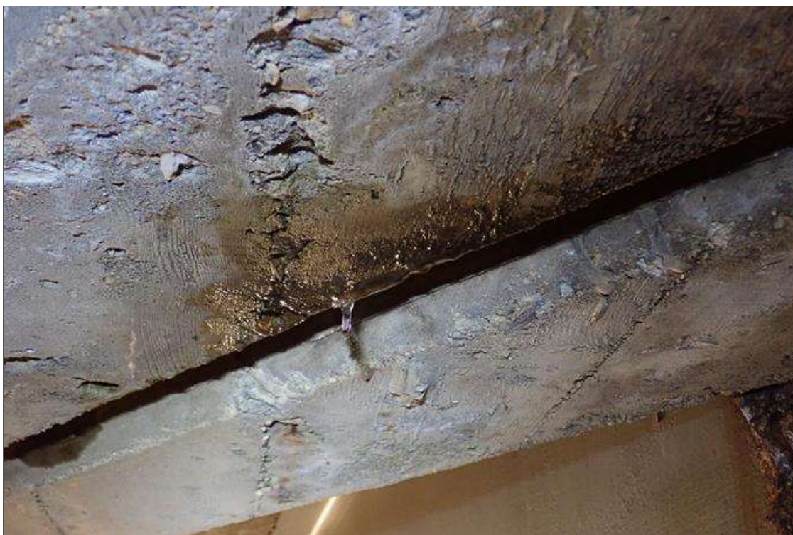
Bent 4 Joint : at random, active dripping
