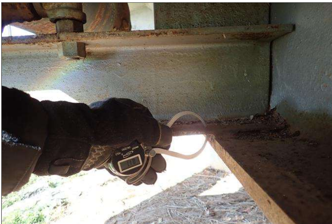
(PAR) right overhang, utility hanger, 7' from end bent 1, bottom flange of bracket at beam, corrosion with section loss (0.2" average remaining x 3")
