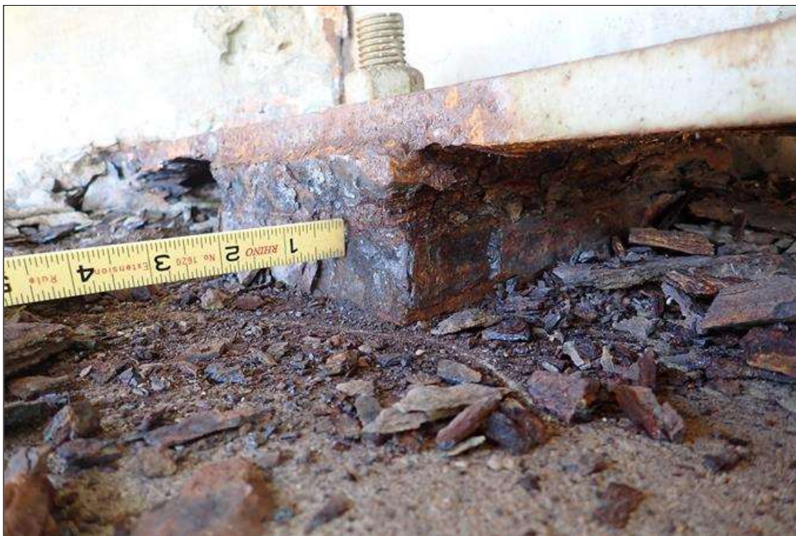
Span 1 Beam 11 Near Bearing 11: (PAR) corrosion with section loss (1/8" loss) at plate edges
