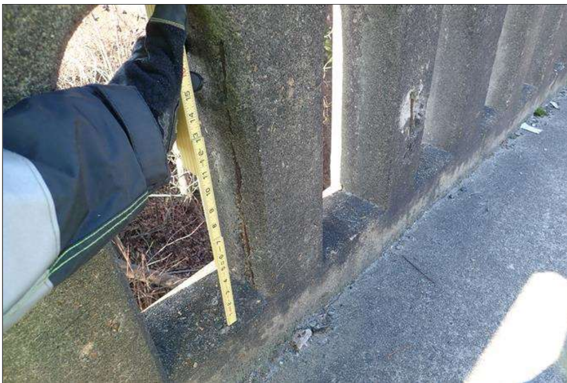
Span 4 Right Bridge Rail: rail posts at random, (4) spalls (up to 16" x 1" x 1/2") with exposed rusted rebar
