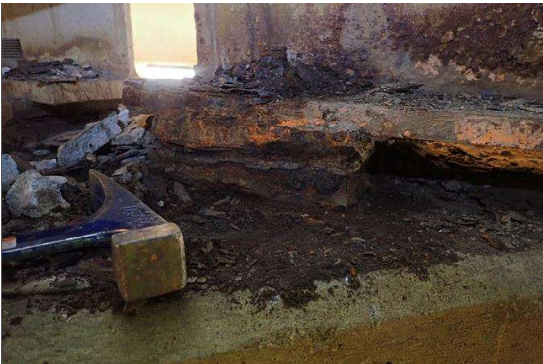
Span 1 Beam 8 Far Bearing 8: (PAR) bearing frozen with pack rust
