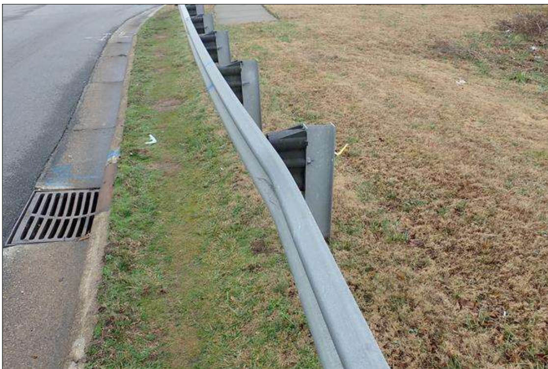
(PAR) southeast guardrail, at center, impact damage (15')
