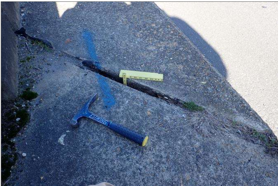
Bent 3 Joint : at right sidewalk, joint material missing (2') with debris and vegetation
