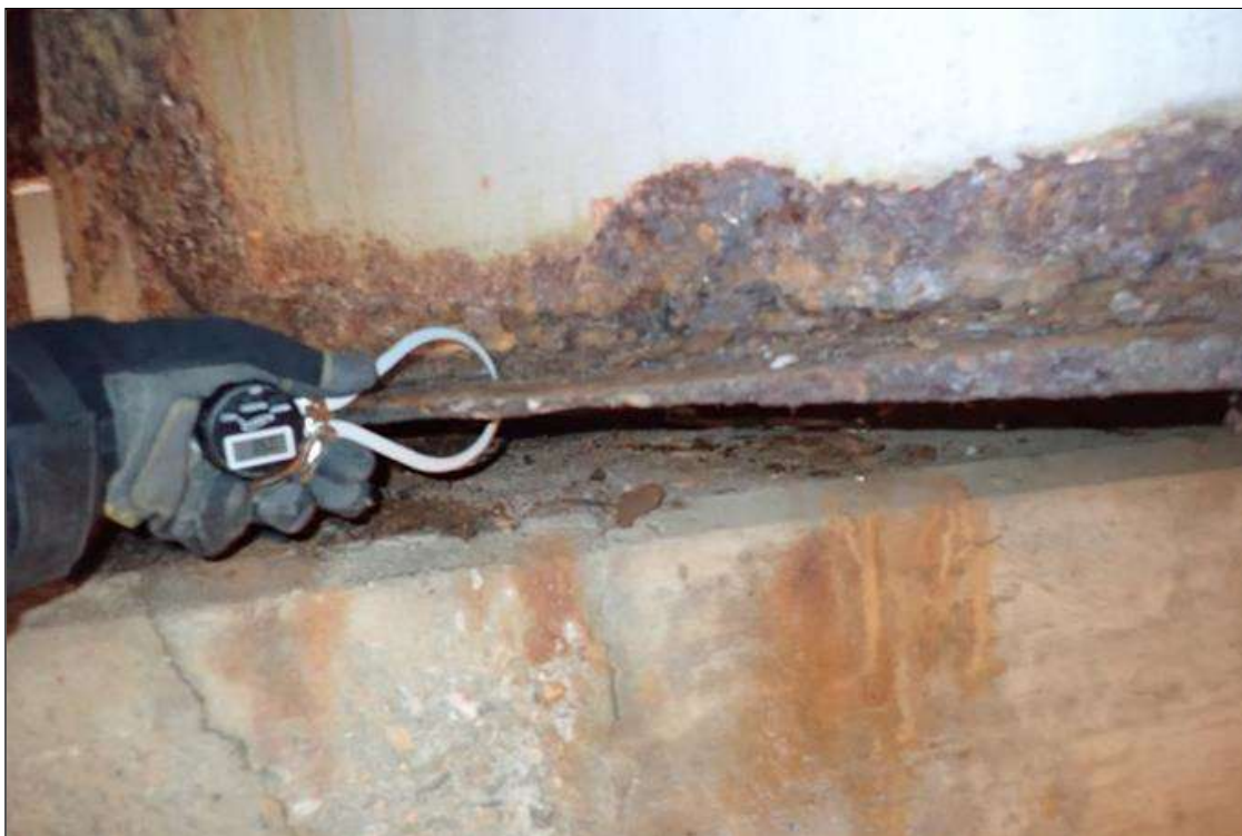
Span 5 Beam 7: (PAR) at bent 4, corrosion with section loss: bottom flange, (0.5" average remaining x 2.5'); web at end diaphragm, (1/4" remaining x 14" x 16"); bottom of web, (5/16" remaining x 3" x 4')
