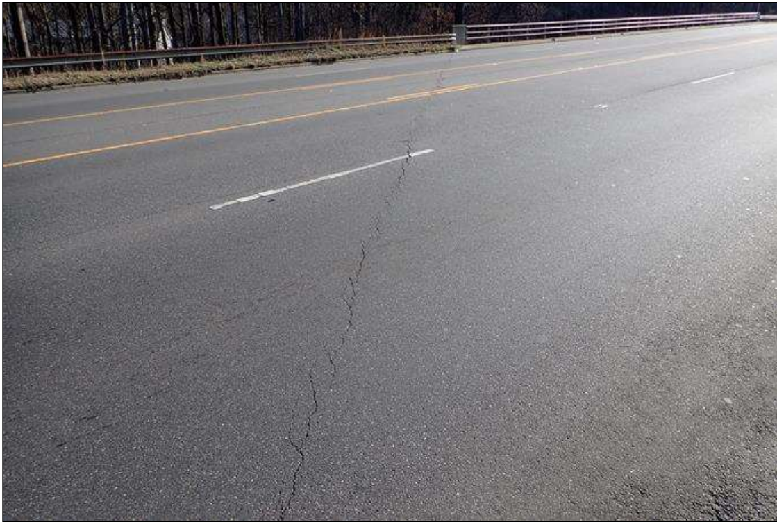
Span 1 Wearing Surface: UP TO 0.25" TRANSVERSE CRACKS IN ASPHALT WEARING SURFACE OVER END BENT 1
