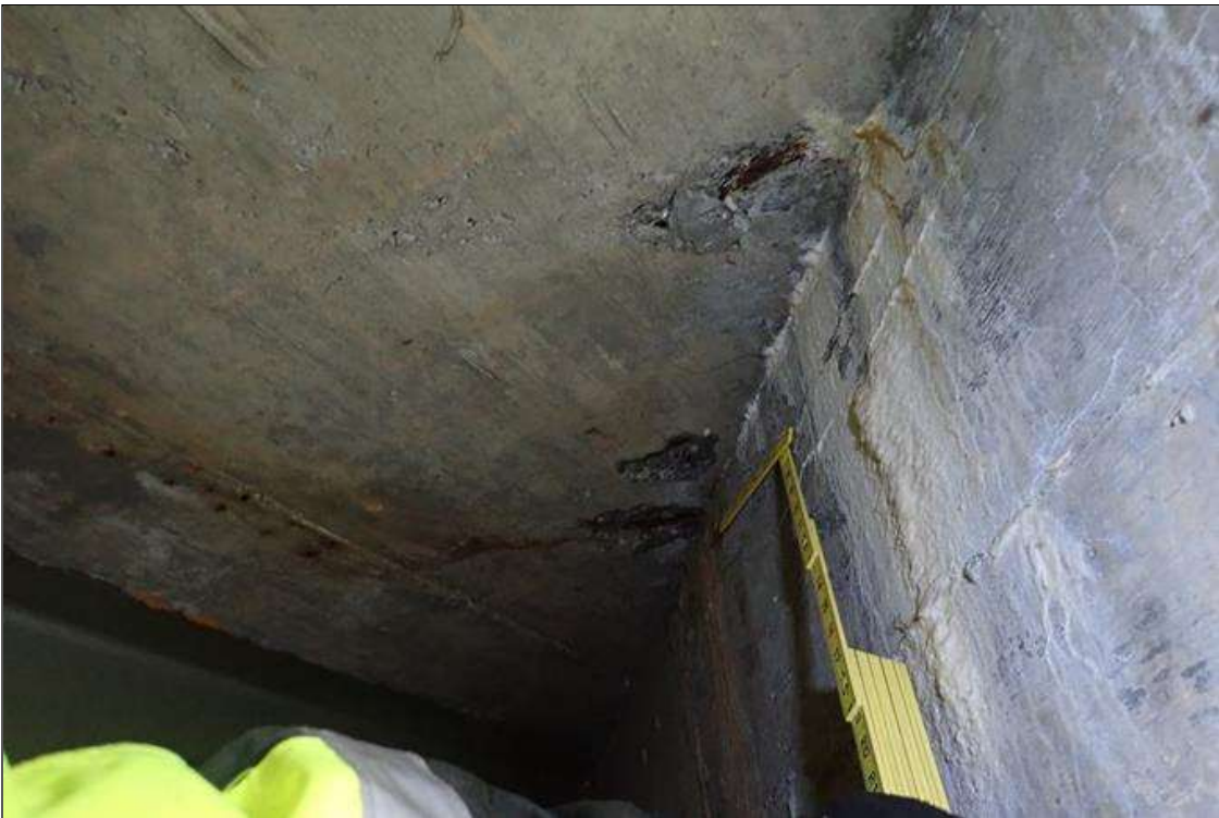
Span 5 Deck: underside, bay 6, at end bent 2, (3) spalls (7" diameter x 1") with exposed rusted rebar
