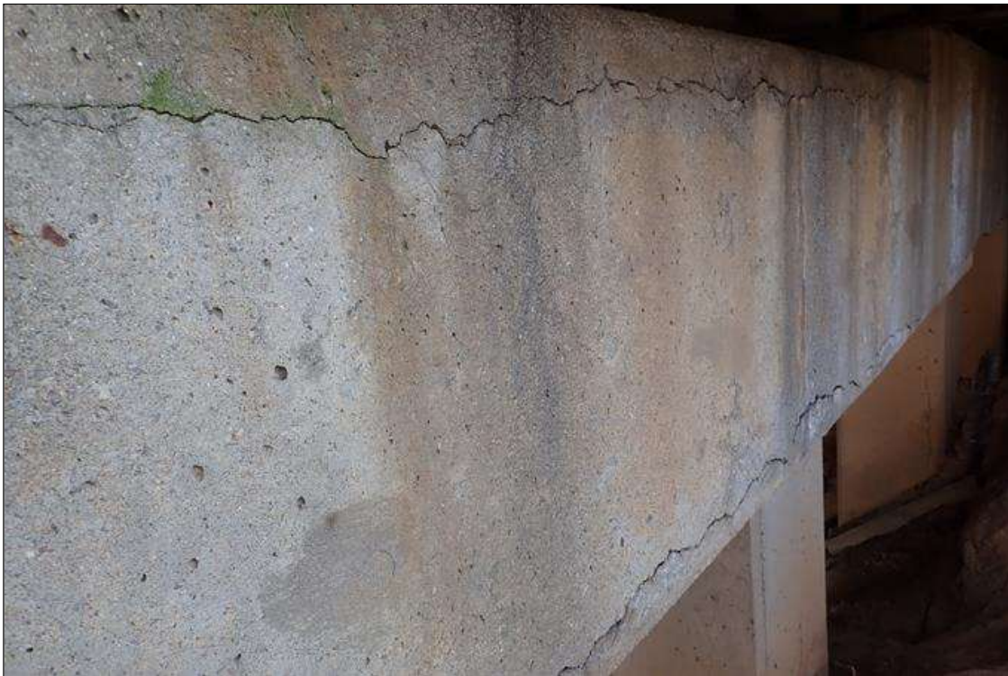
Bent 4 Cap 1: (PAR) span 5 face, from beam 8 to 11, longitudinal cracks (1/8" x 30') at top and bottom corners with delamination (up to full height x 30') and spalls (19' x up to 20" x 2") with exposed rusted rebar; cracks and delamination similar on span 4 face
