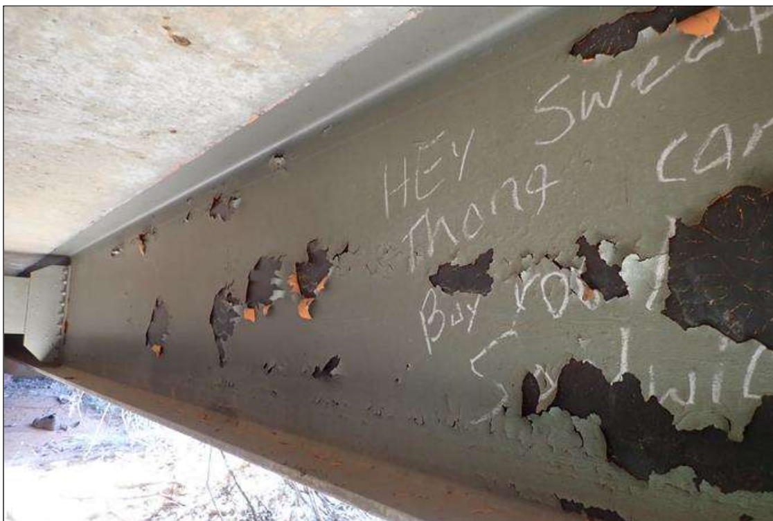
Span 5 Beam 11: paint peeling at random
