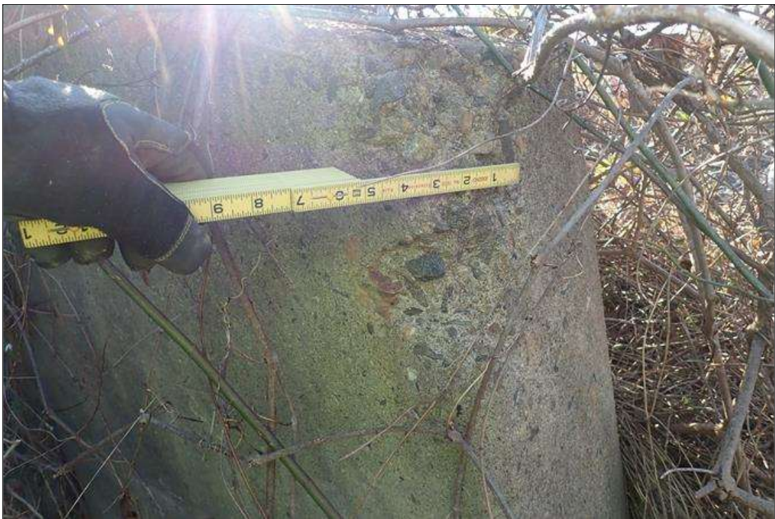
southeast wingwall, at end, spall (6" x 4" x 1")
