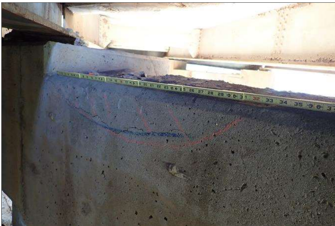
Bent 1 Cap 1: span 1 face, bay 9, top corner, delamination (2.5' x 6")
