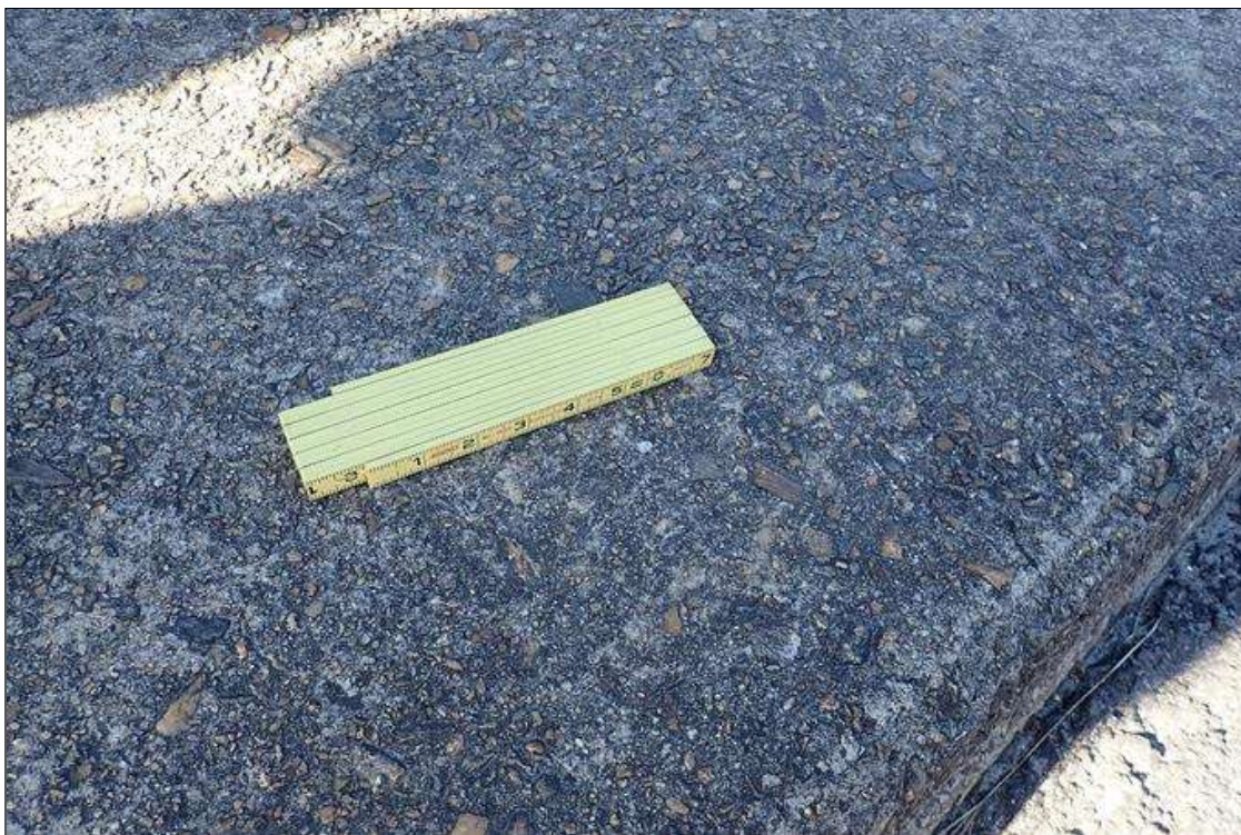
Span 4 Right Bridge Rail: throughout sidewalk and rail, scale with secure aggregate
