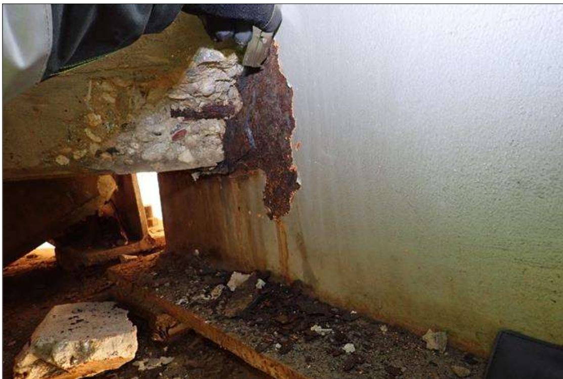
Span 1 Beam 10: (PAR) at bent 1, left face of web, corrosion with section loss (3/8" remaining x 7" x 8")
