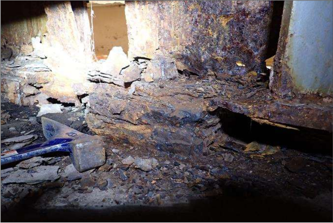
Span 1 Beam 7 Far Bearing 7: (PAR) bearing frozen with pack rust
