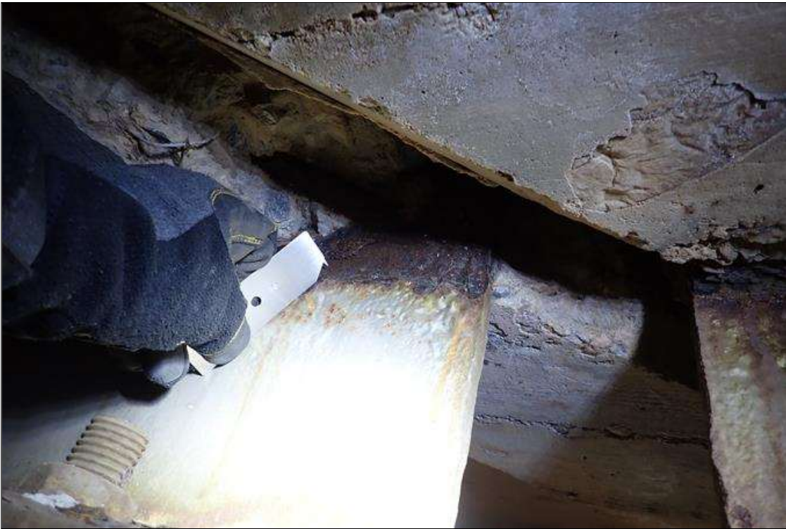
Span 2 Beam 8: (PAR) at bent 1, web at end diaphragm, corrosion with section loss (5/16" remaining x 10" x 7")
