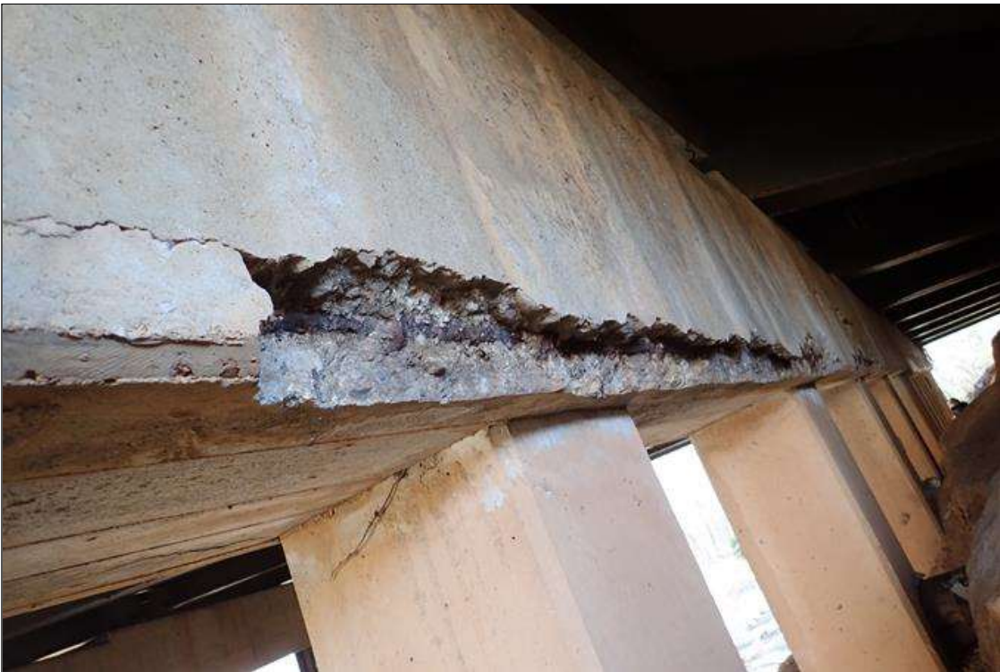
Bent 4 Cap 1: (PAR) span 5 face, from beam 8 to 11, longitudinal cracks (1/8" x 30') at top and bottom corners with delamination (up to full height x 30') and spalls (19' x up to 20" x 2") with exposed rusted rebar; cracks and delamination similar on span 4 face
