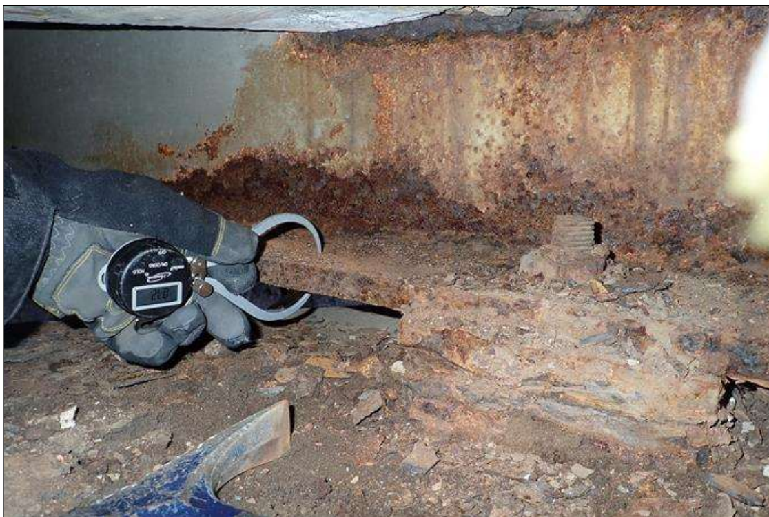
Span 2 Beam 9: (PAR) at bent 1, corrosion with section loss: bottom flange, (0.7" average remaining x 1.5'); web, at end diaphragm, (1/16" remaining x 16" x 4") with corrosion hole (1.5" x 1/2")
