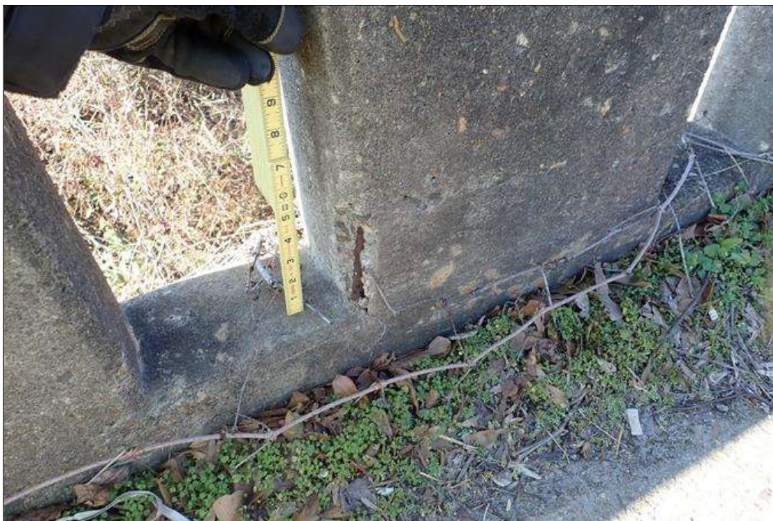
Span 5 Right Bridge Rail: rail post at random, (3) spalls (up to 5" x 2" x 1/2") with exposed rusted rebar
