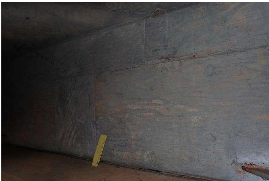
End Bent 2 Abutment/Backwall : bay 1, multiple vertical and diagonal cracks (1/32" x 3')
