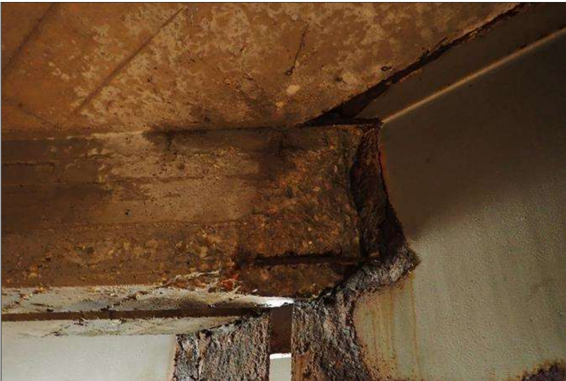
Span 5 Deck: bent 4 end diaphragm, bay 7 at beam 7, spall (2' x 18" x 2") with exposed rusted rebar
