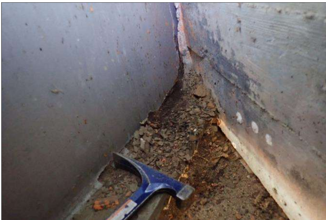
Span 1 Beam 9: at end bent 1, bottom of web, corrosion with section loss (7/16" remaining x 3" x 1')
