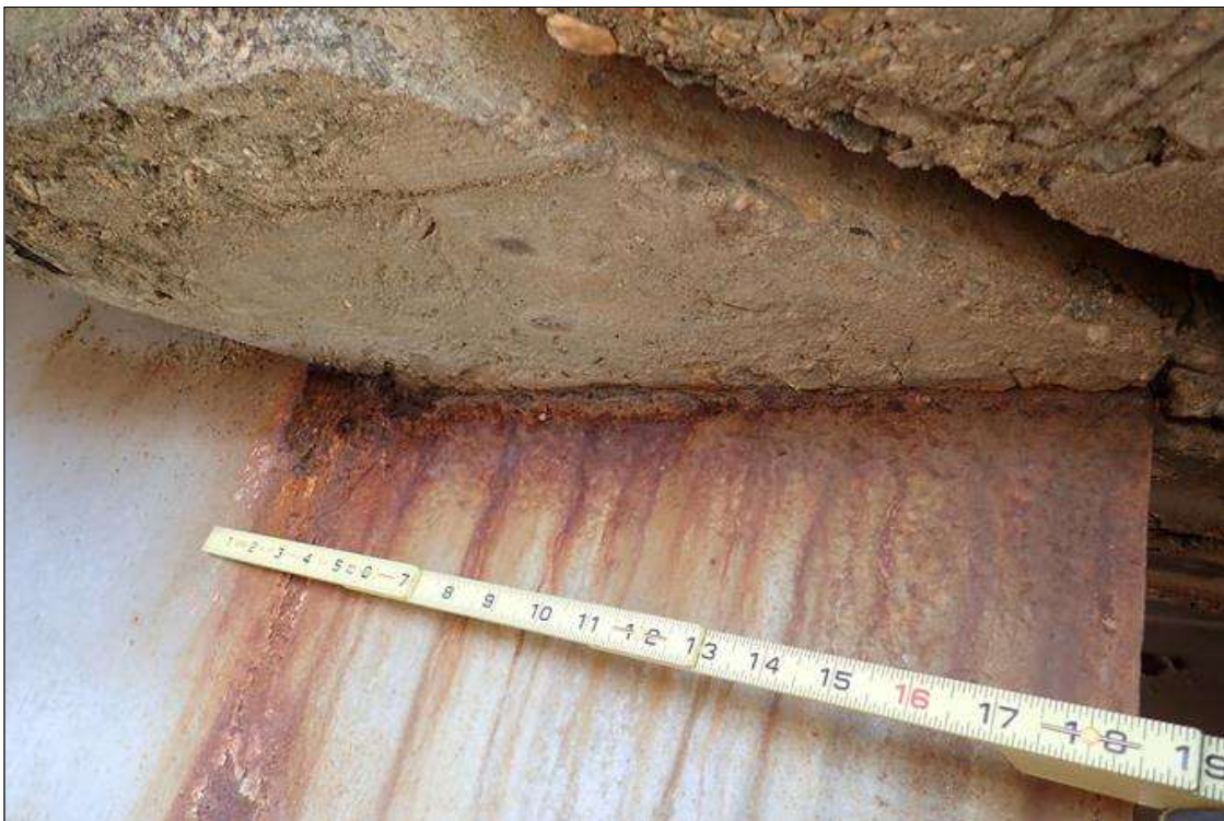
Span 4 Beam 11: (PAR) at bent 4, corrosion with section loss: web at end diaphragm, (1/4" remaining x 10" x 4")
