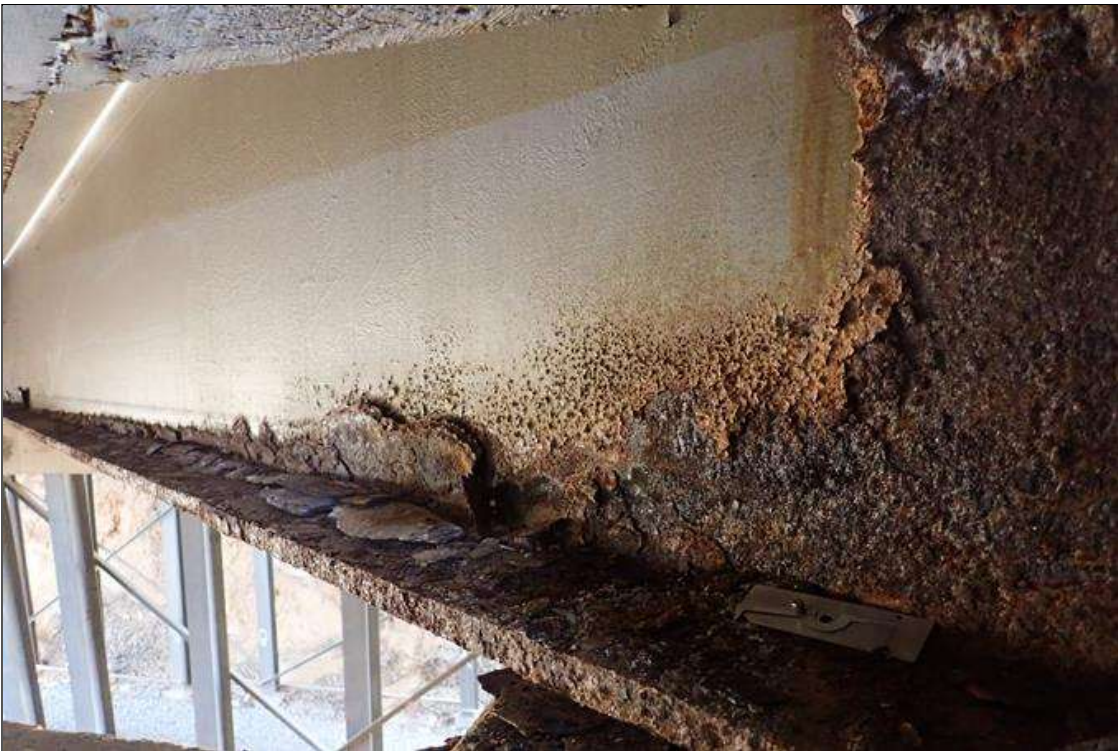
Span 4 Beam 7: (PAR) at bent 4, corrosion with section loss: web, at bearing, (3/8" remaining x 16" x 12"); bottom of web, (1/4" remaining x 2" x approximately 15'); bottom flange, (0.7" average remaining x 16")
