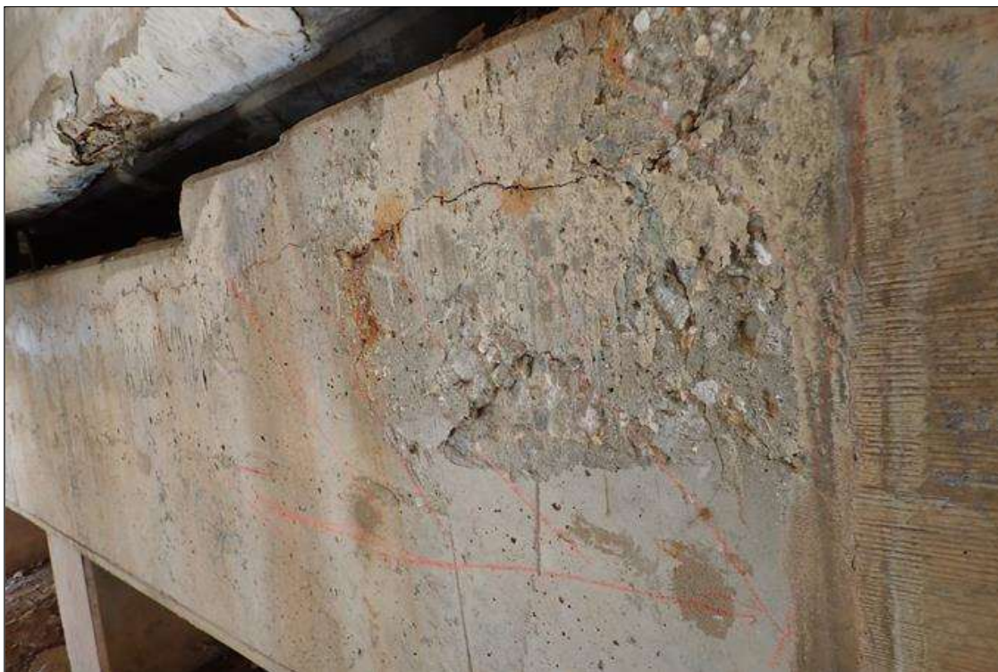
Bent 1 Cap 1: span 2 face, below beams 7 - 11, longitudinal crack (1/8" x 48') with areas of delaminations/spalls (up to 2' high x 1/2" deep), with some rust stains
