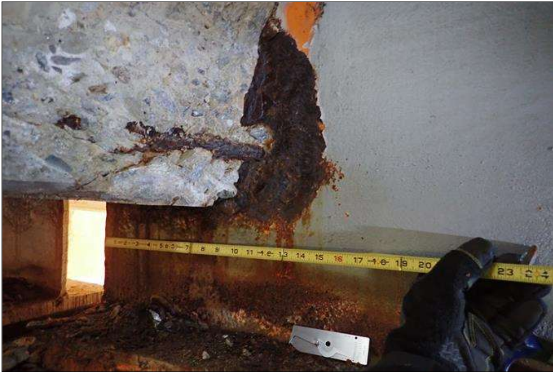
Span 1 Beam 8: (PAR) at bent 1 end diaphragm, web, corrosion with section loss (1/16" remaining x 16" x 10"); bottom flange, rust scale
