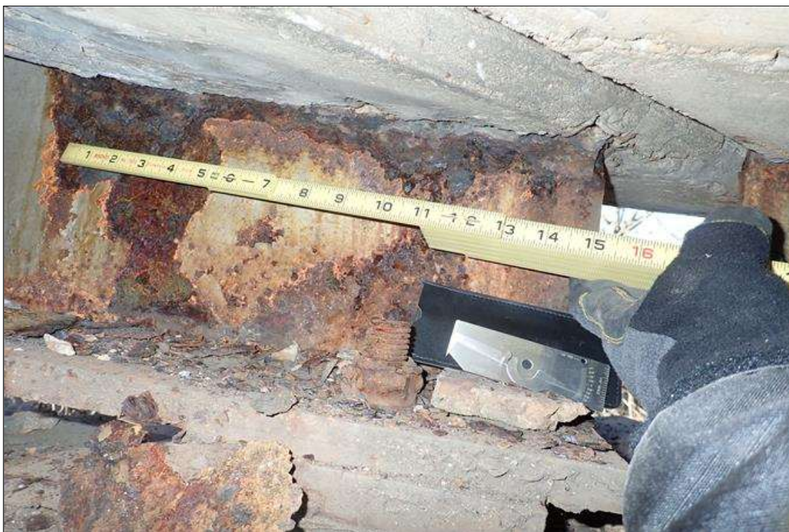
Span 2 Beam 11: (PAR) at bent 1, corrosion with section loss: web at end diaphragm, (0.25" remaining x 16" x 2")
