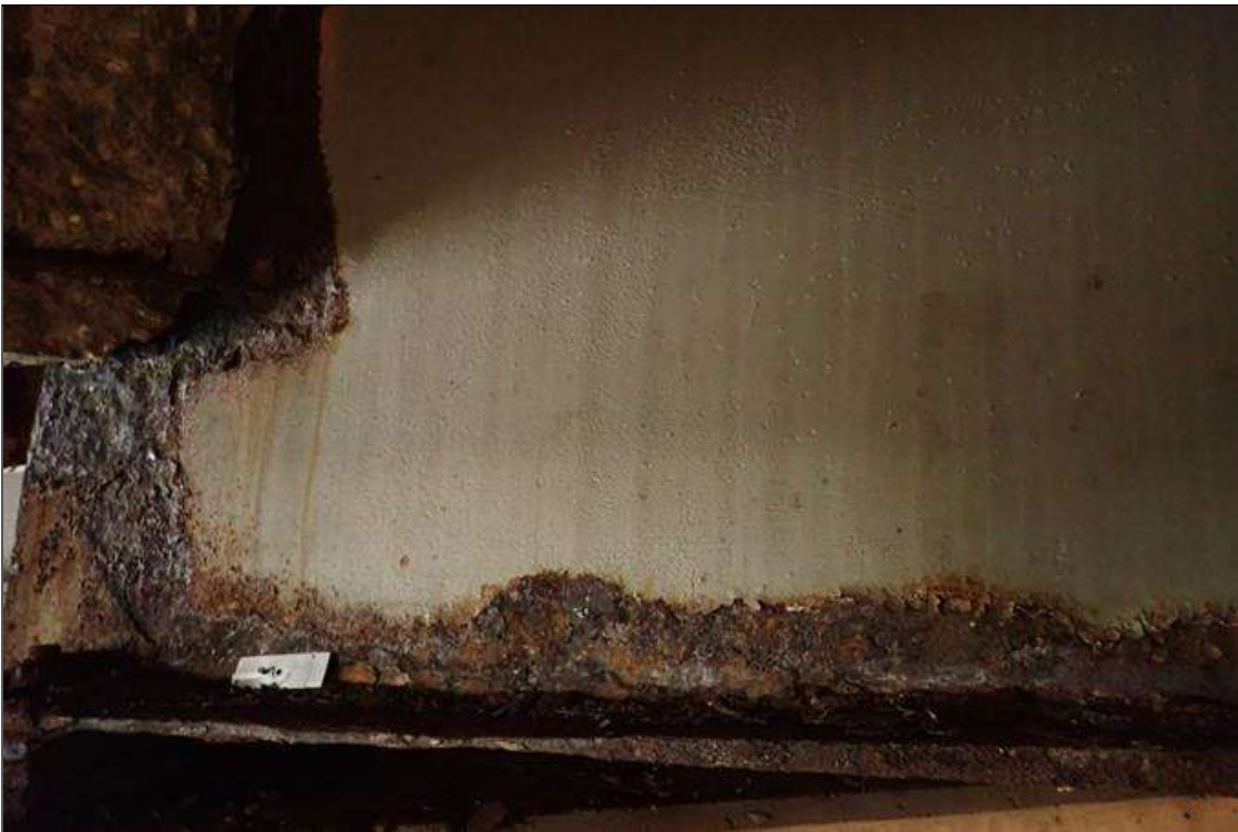
Span 5 Beam 7: (PAR) at bent 4, corrosion with section loss: bottom flange, (0.5" average remaining x 2.5'); web at end diaphragm, (1/4" remaining x 14" x 16"); bottom of web, (5/16" remaining x 3" x 4')
