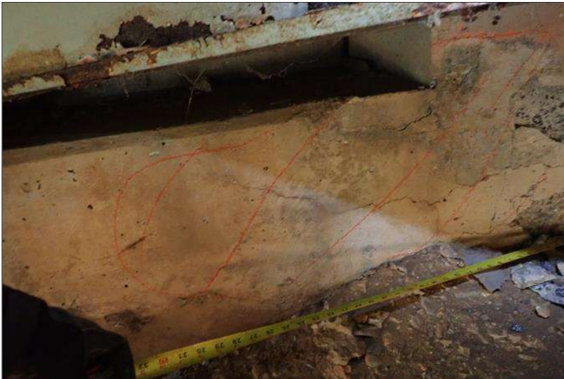
End Bent 1 Cap 1: face of cap, below beam 7, spall/delamination (3.5' x 1.5' x 1")
