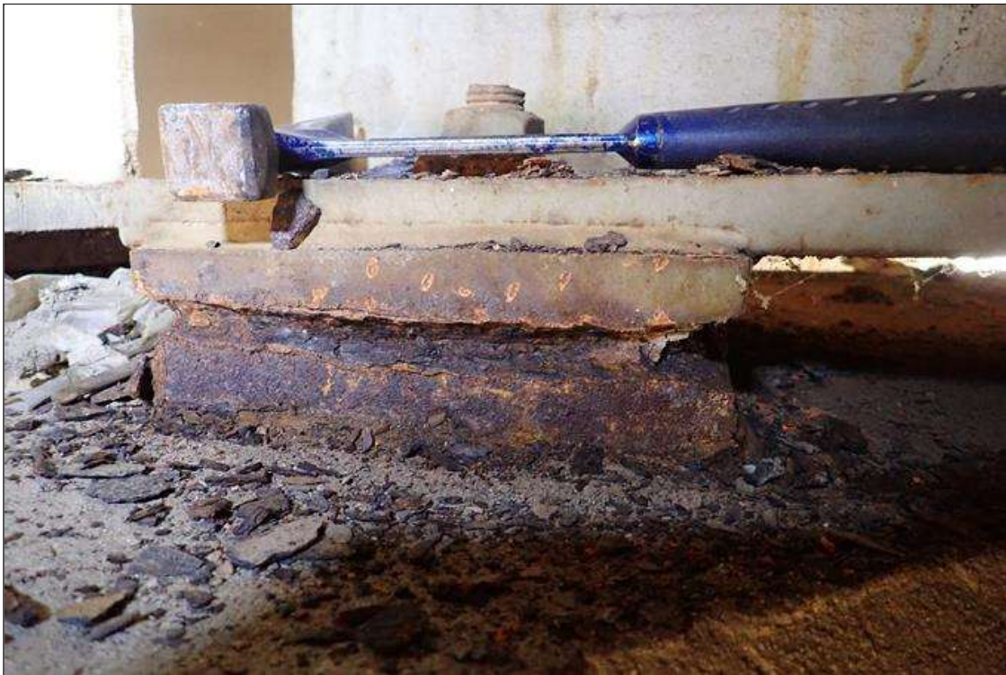
Span 5 Beam 8 Near Bearing 8: (PAR) bearing frozen with pack rust
