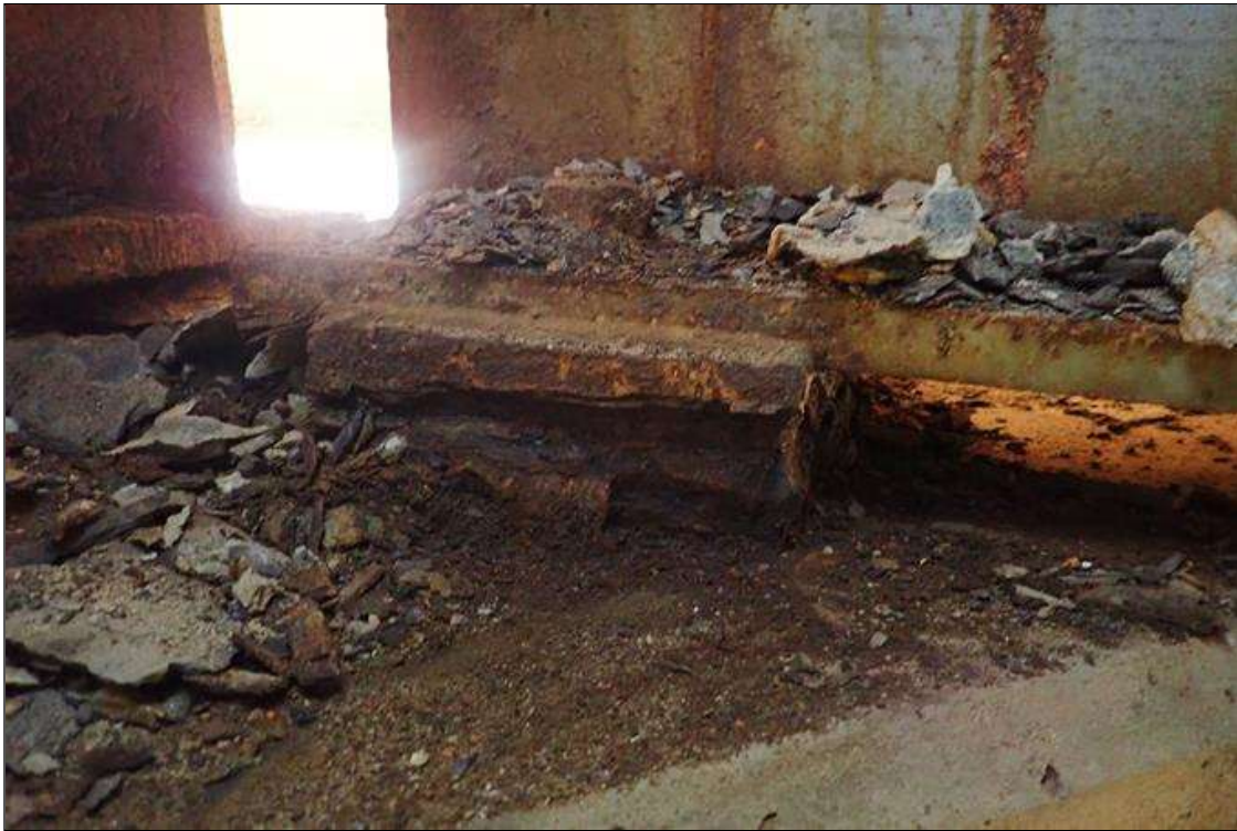
Span 1 Beam 9 Far Bearing 9: (PAR) bearing frozen with pack rust
