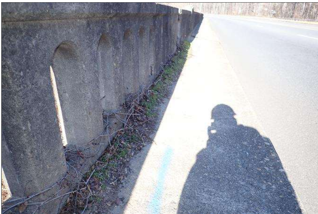
Span 5 Right Bridge Rail: along top of sidewalk, vegetation (1' wide x 20')
