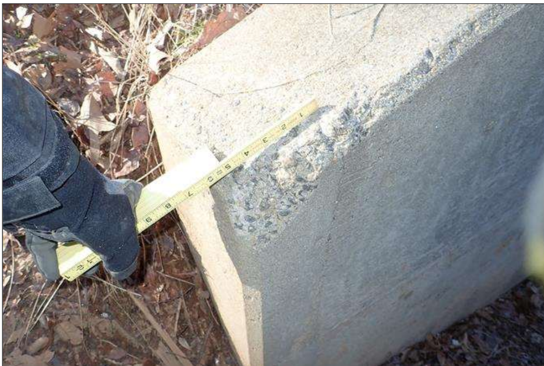
northeast wingwall, top corner at end, spall (6" x 3" x 1/2")
