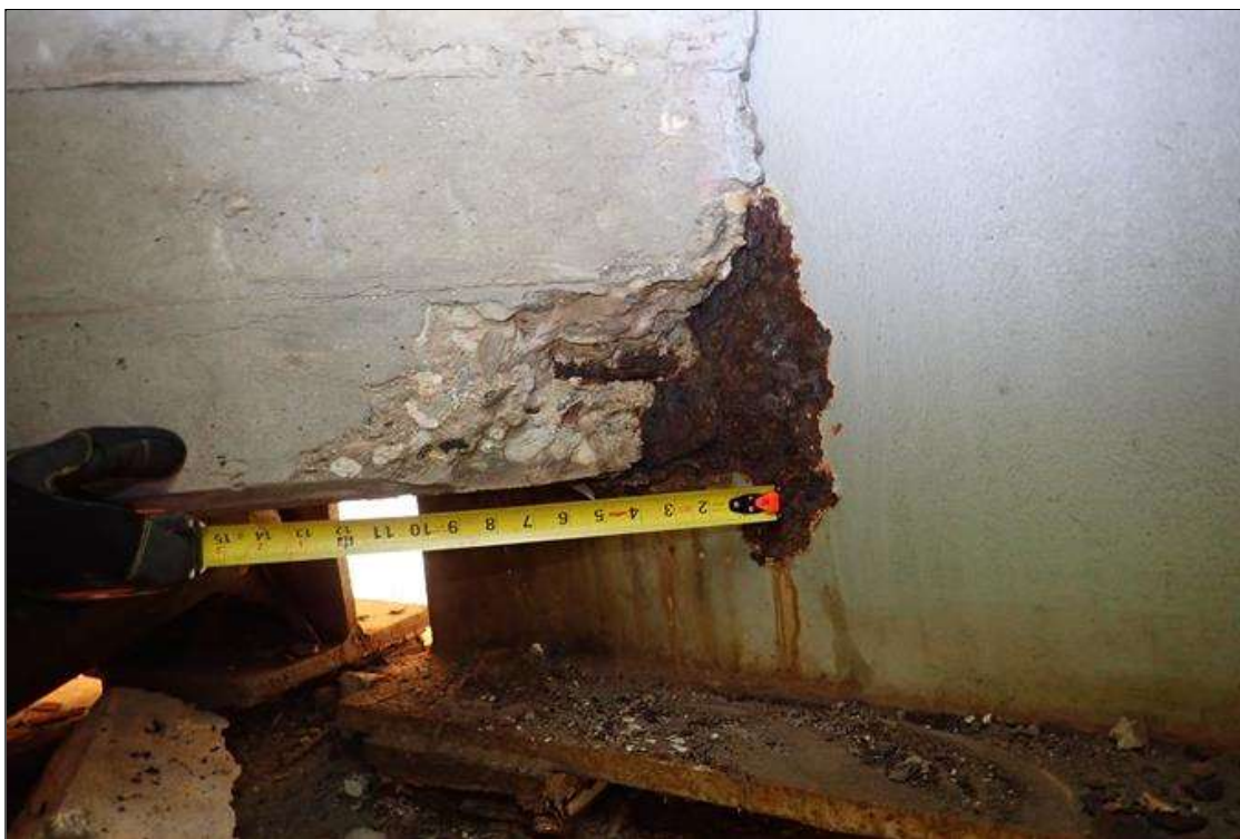
Span 1 Deck: bent 1 end diaphragm, bay 9. at beam 10, spall (12" x 6" x 6") with exposed rusted rebar
