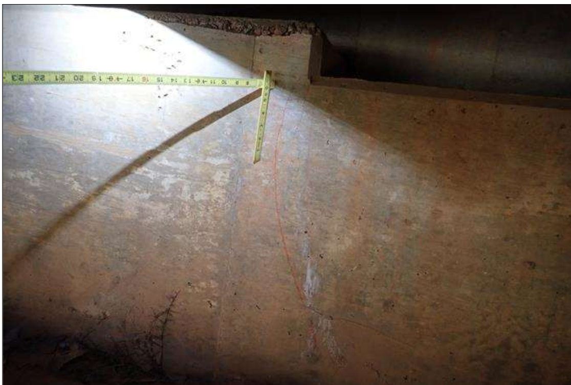
End Bent 2 Cap 1: at random, vertical cracks (hairline x up to 2') with efflorescence
