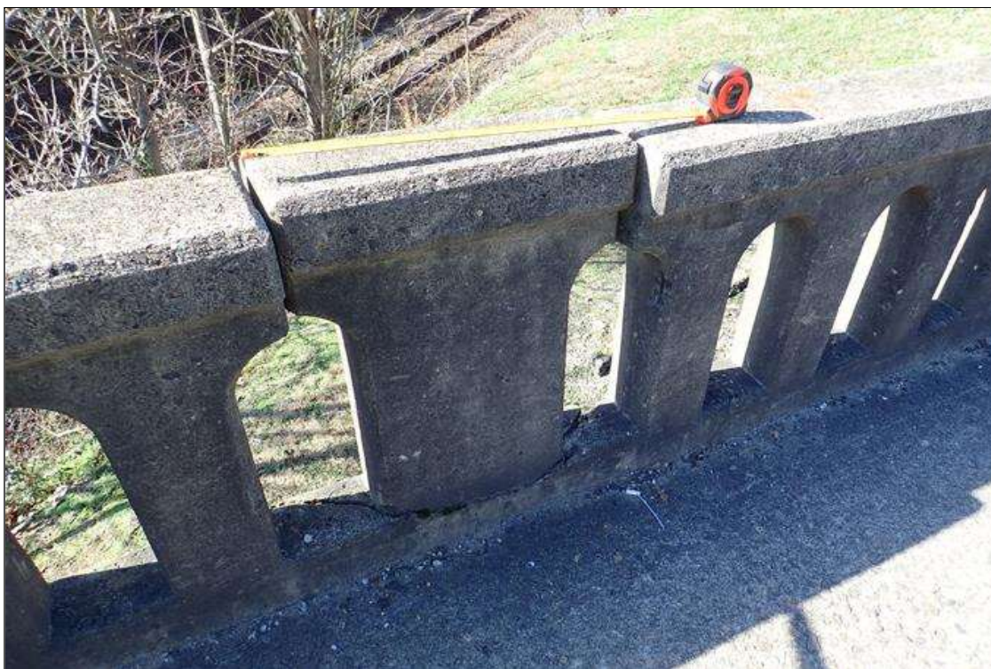
Span 1 Right Bridge Rail: (PAR) at midspan, impact damage (2'), broken at base
