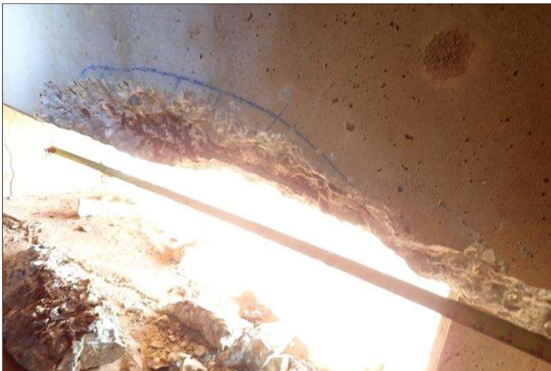
Bent 1 Cap 1: (PAR) span 1 face, below bay 9, bottom corner, spall (5' x 8" x 3") with exposed rusted rebar
