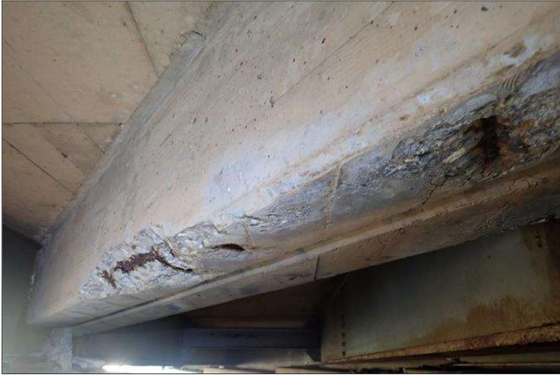
Span 2 Deck: bent 1 end diaphragm, bay 9, (2) spalls (up to 3.5' x 8" x 3") with exposed rusted rebar
