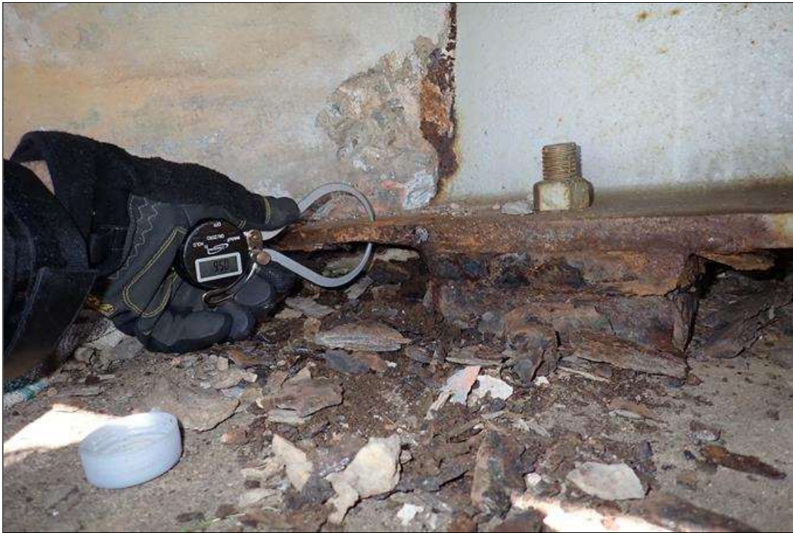
Span 1 Beam 11: (PAR) at end bent 1, behind bearing, corrosion with section loss (0.6" average remaining x 1')
