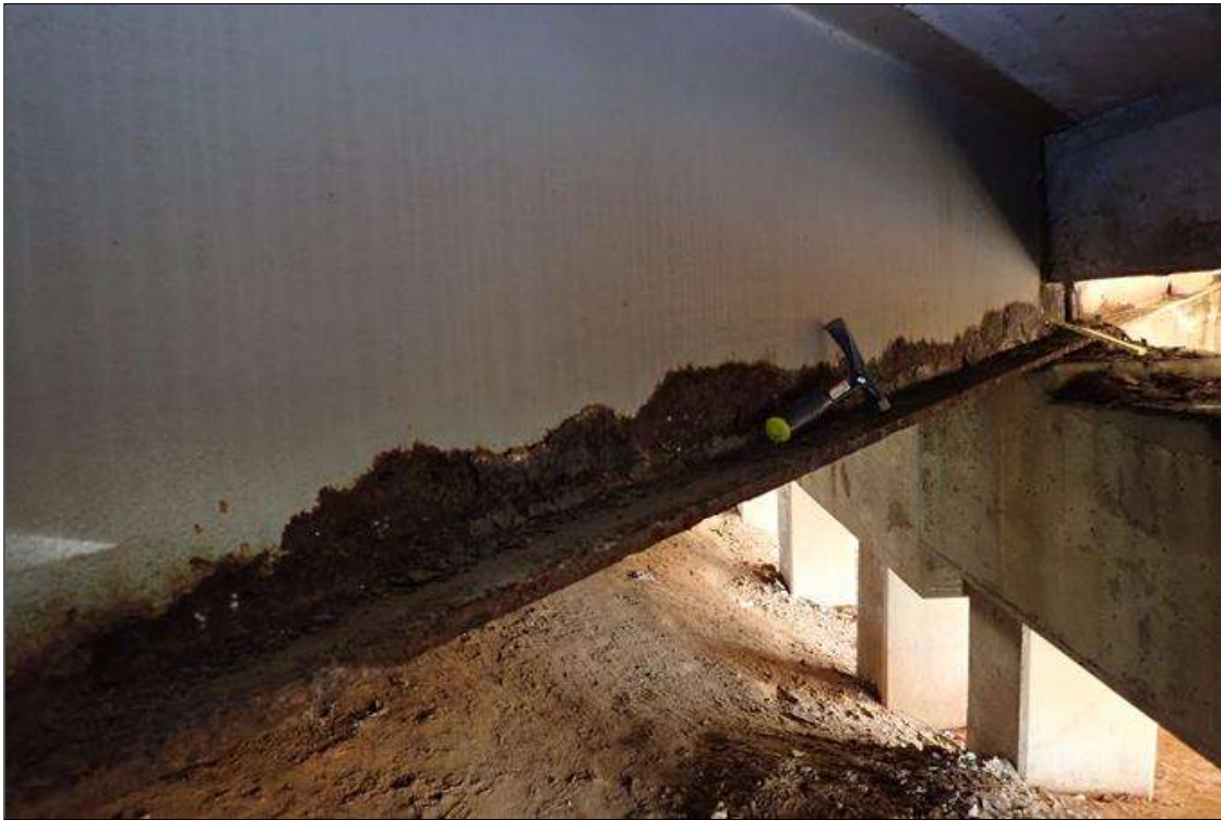
Span 1 Beam 7: (PAR) at bent 1, corrosion with section loss: web, corrosion hole at bearing (12" x 3"); bottom of web, (1/8" remaining x 4" x 11'), (5/16" remaining x 1" x next 6')
