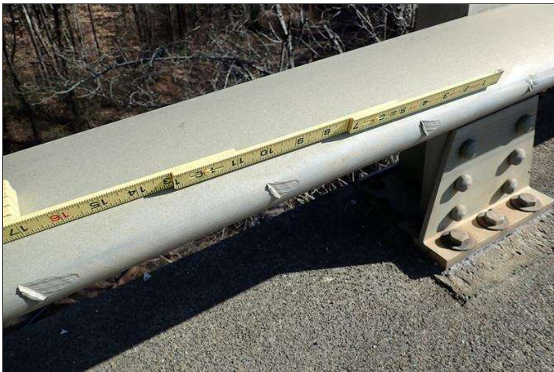
Span 4 Left Bridge Rail: at bent 4, bottom rail, impact damage with gouges (1/8" deep x 4')
