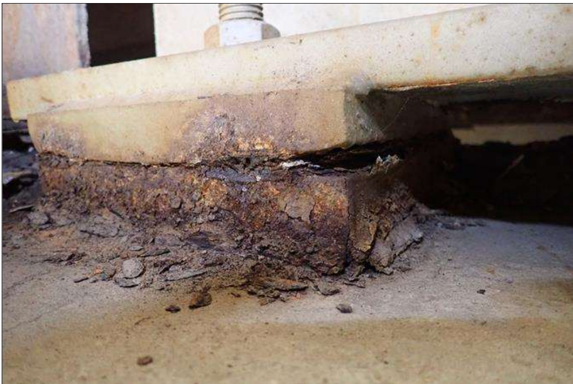
Span 2 Beam 8 Near Bearing 8: pack rust
