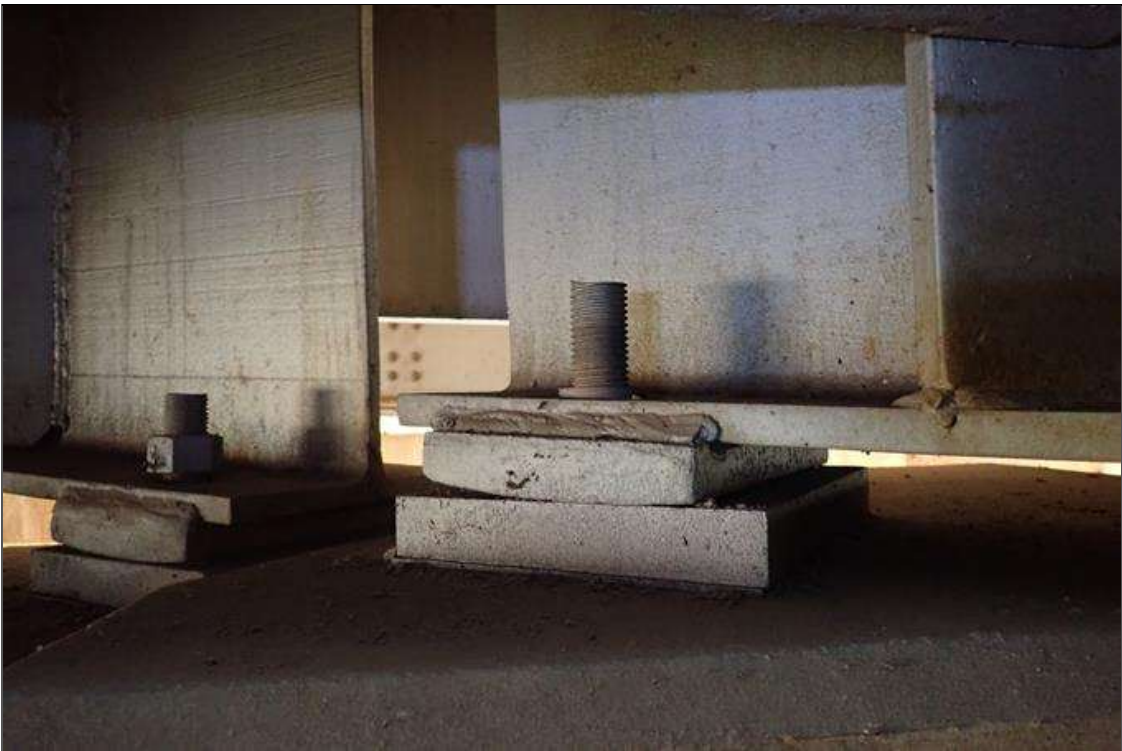
Span 1 Beam 5 Far Bearing 5: left anchor bolt nut missing
