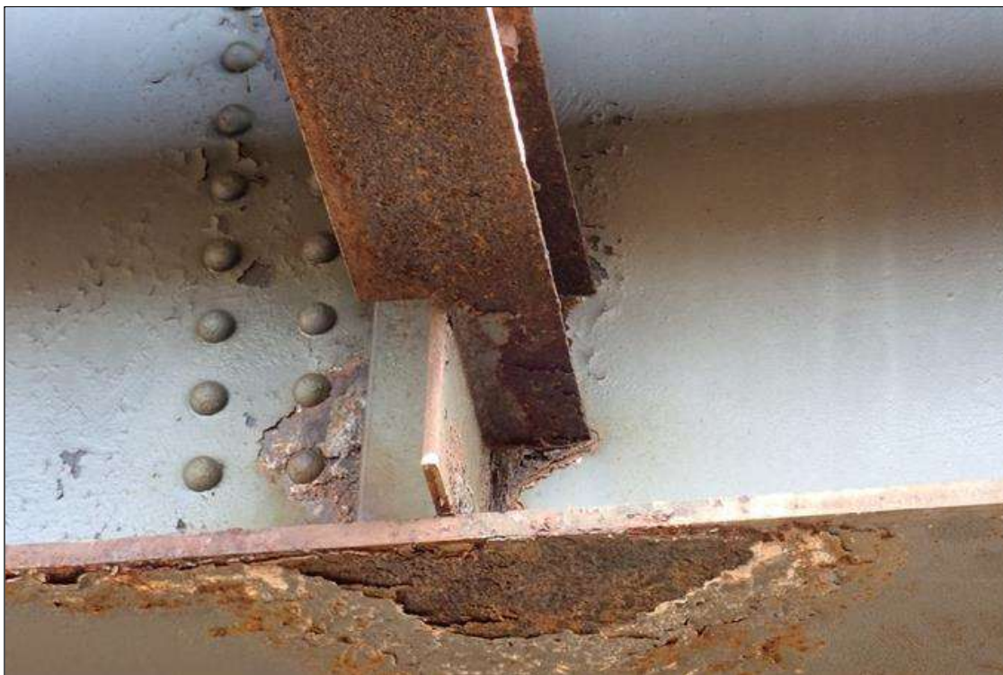
Span 4 Beam 11: midspan at utility connection, rust scale (no ladder access to verify remaining section)
