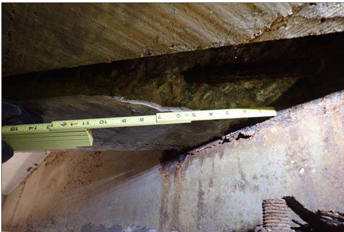
Span 2 Deck: bent 1 end diaphragm, bay 9, at beam 10, spall (18" x 4" x 2") with exposed rusted rebar
