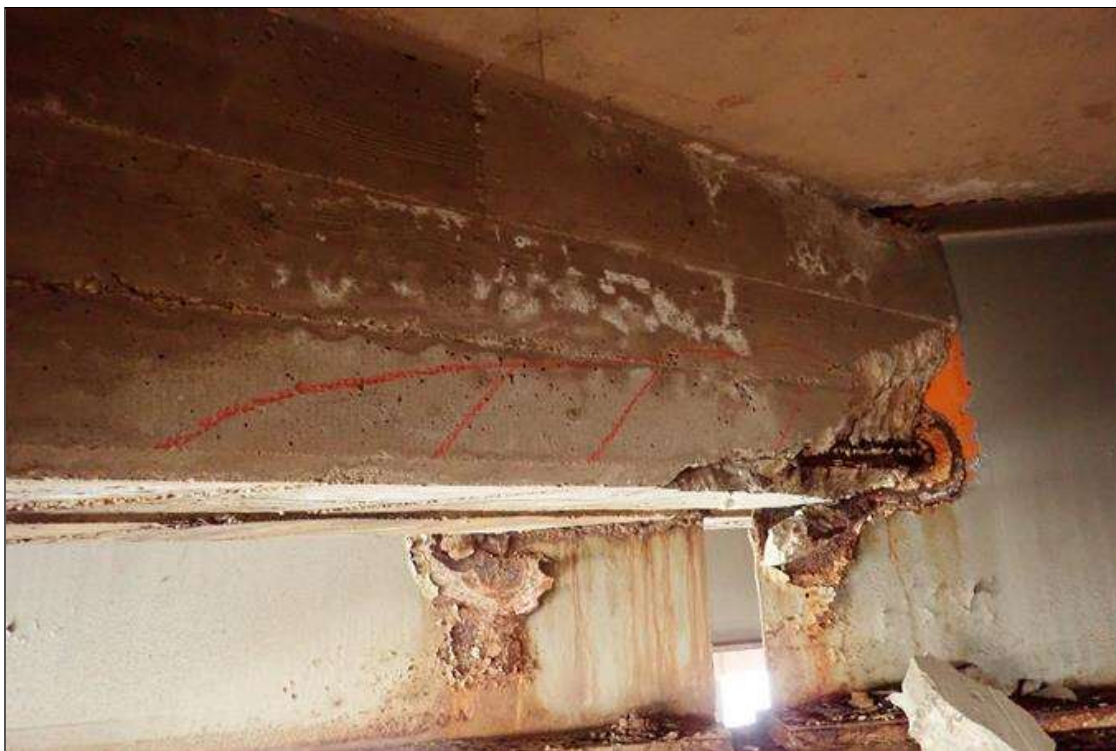
Span 5 Deck: bent 4 end diaphragm, bay 9, at beam 9, delamination/spall (4' x 1' x 3") with exposed rusted rebar
