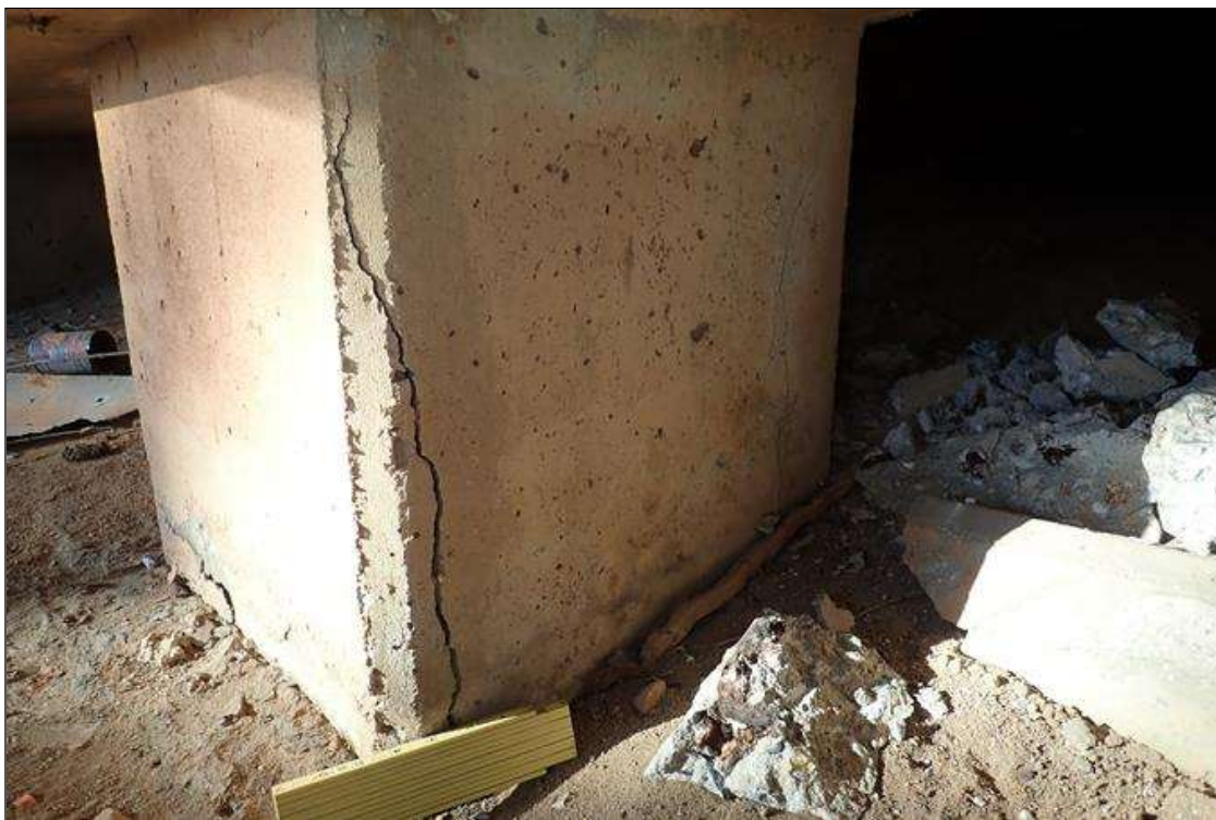
Bent 1 Pile 13: vertical cracks (up to 1/4" x 2')
