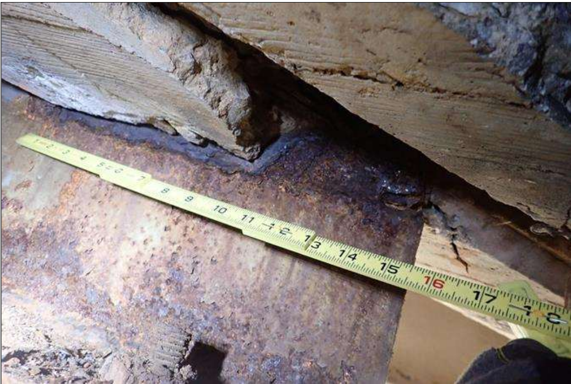
Span 2 Beam 9: (PAR) at bent 1, corrosion with section loss: bottom flange, (0.7" average remaining x 1.5'); web, at end diaphragm, (1/16" remaining x 16" x 4") with corrosion hole (1.5" x 1/2")
