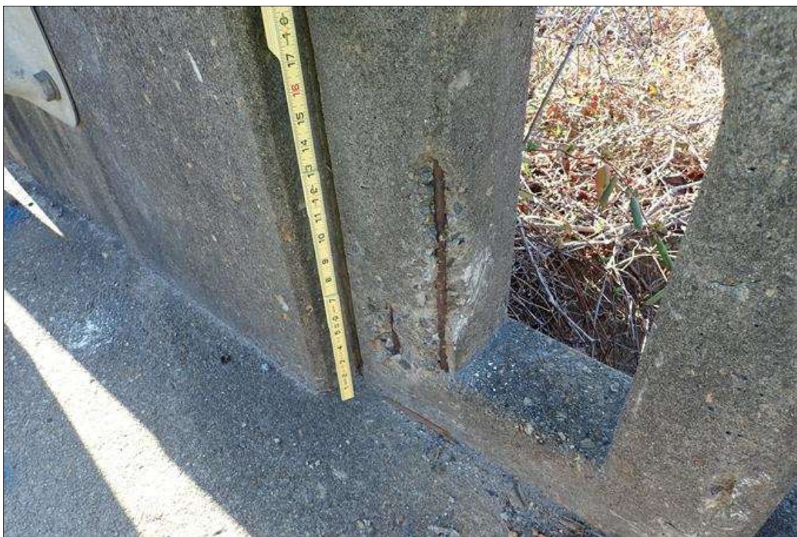
Span 5 Right Bridge Rail: at end bent 2, rail post, spall (12" x 5" x 1") with exposed rusted rebar
