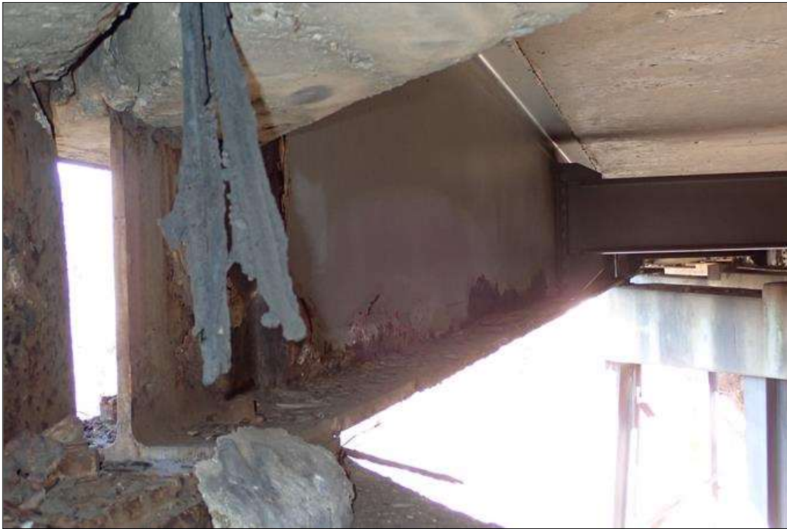
Span 4 Beam 11: 2020 no ladder access to verify section remaining, previously noted as: BEAM 11 SPAN 4 AT BENT 4: SECTION LOSS TO BOTTOM LEFT FLANGE WITH 11/16" REMAINING AND BOTTOM 4" OF WEB WITH 7/16" REMAINING FOR 15'
