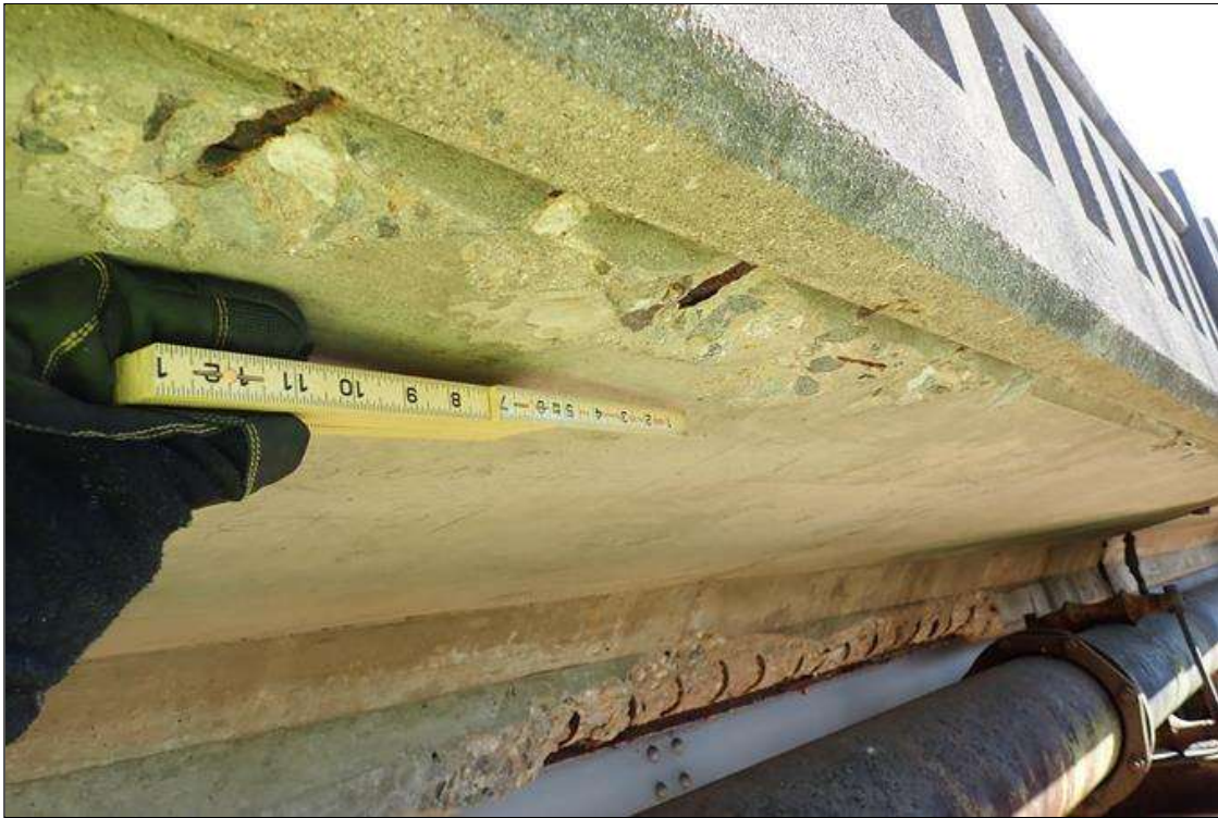
Span 1 Deck: along right drip edge, multiple spalls (up to 2' x 4" x 1/2") with exposed rusted rebar
