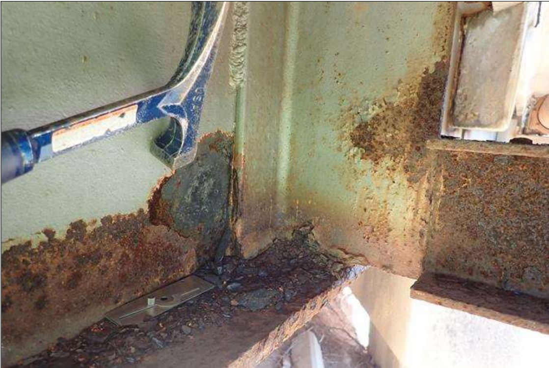
Span 1 Beam 11: (PAR) 8' from bent 1, at utility hanger, right face of web, corrosion with section loss (1/8" remaining x 6" x 6")
