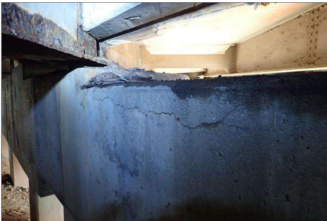
Bent 1 Cap 1: span 1 face, below beam 7, longitudinal crack (1/16" x 3')
