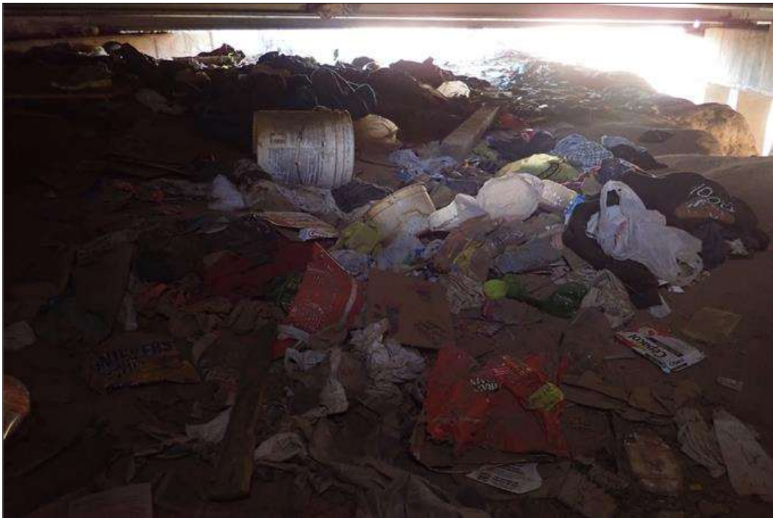
limited access to right half of span 5 due to vagrant debris
