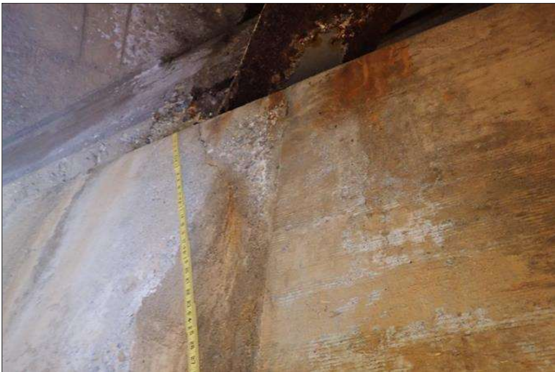
Bent 4 Cap 1: span 5 face at beam 7, vertical crack (1/16" x 2') with efflorescence
