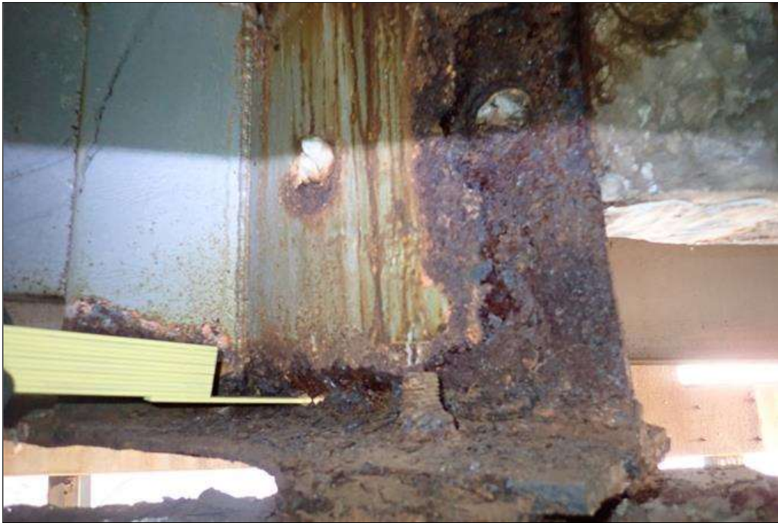
Span 2 Beam 7: (PAR) at bent 1, corrosion with section loss: bottom flange, (0.6" average remaining x 3'); web at bearing, (1/16" remaining x 1' x 16" high) with corrosion hole (2" x 1")
