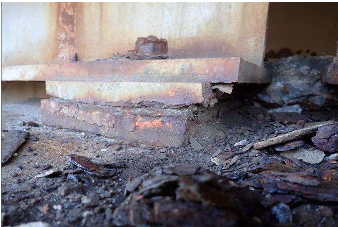
Span 4 Beam 11 Far Bearing 11: pack rust
