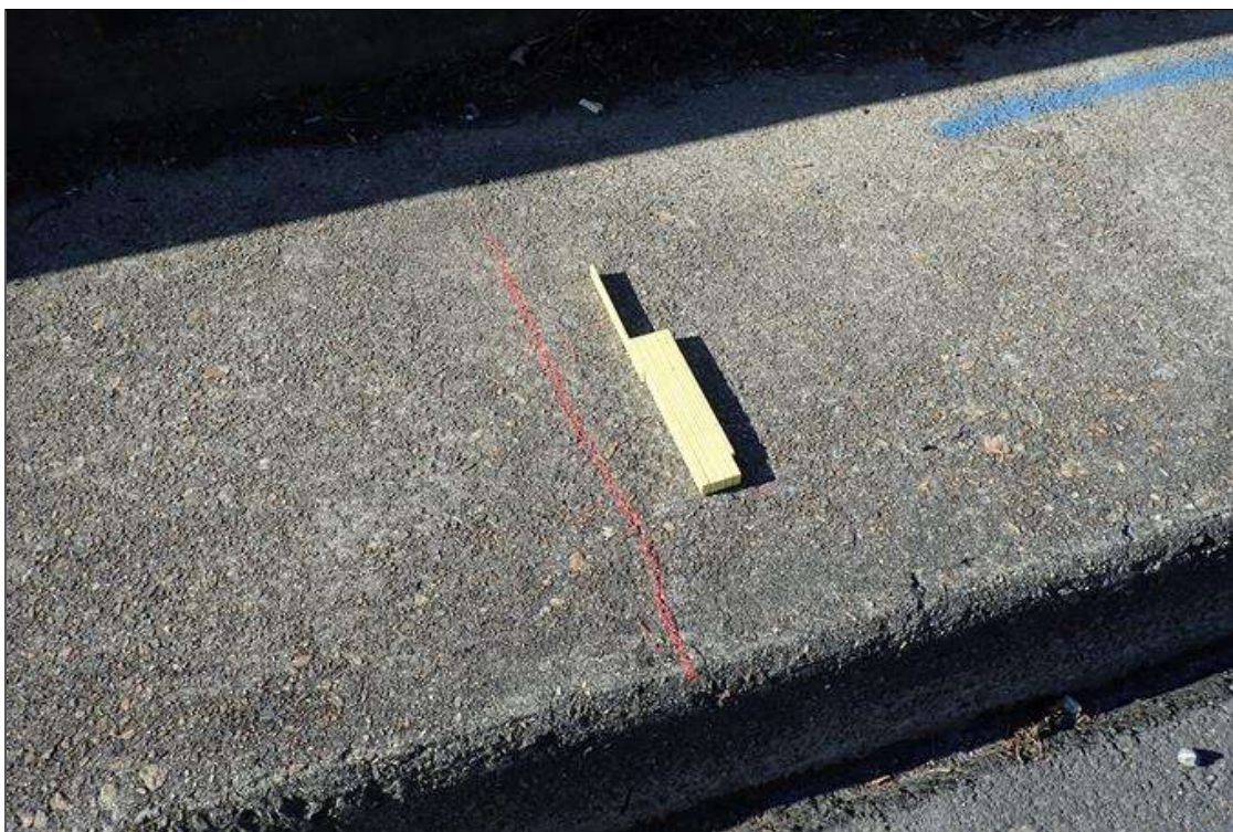
Span 5 Right Bridge Rail: at midspan, sidewalk, transverse crack (1/32" x 3')
