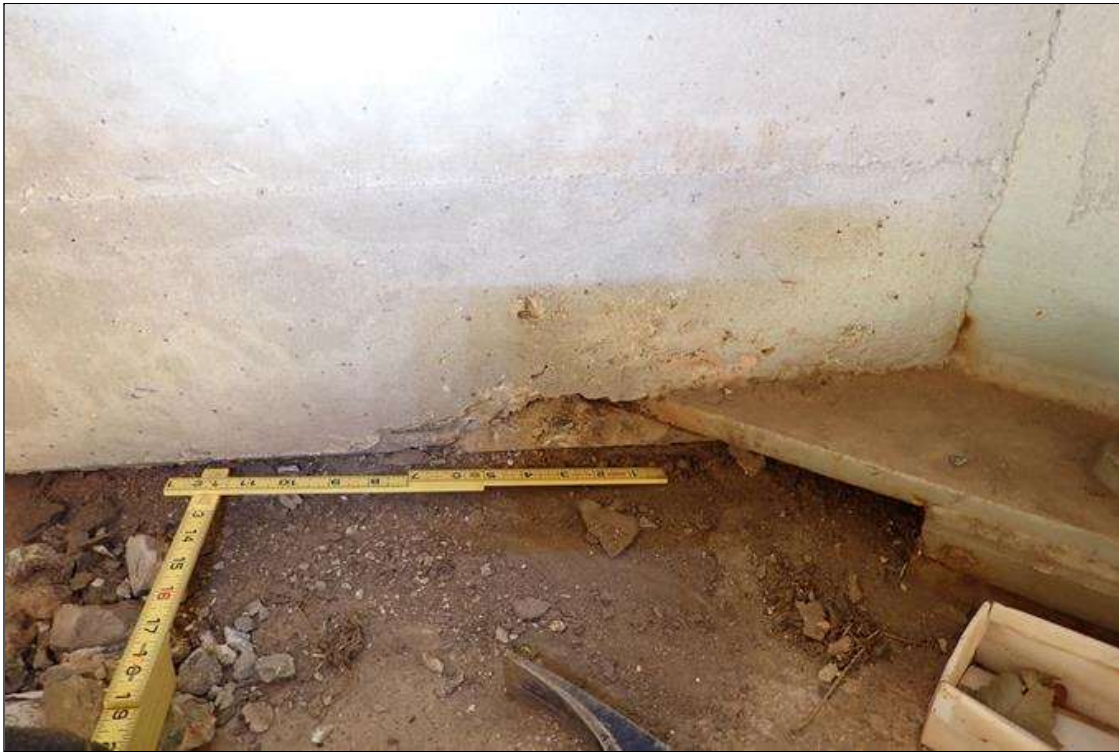
End Bent 1 Abutment/Backwall : bay 9 at beam 10 bottom flange, spall (8" x 2" x 1")
