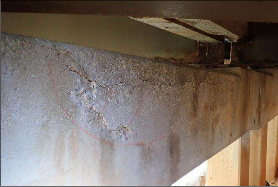
Bent 4 Cap 1: span 5 face, bay 7, delamination/spall (7' x 20" x 1") with longitudinal crack (1/8"); similar span 4 face
