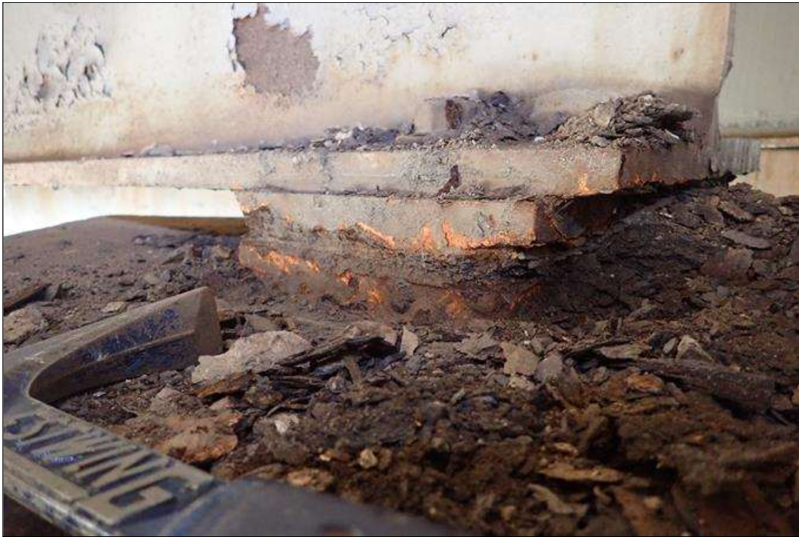
Span 4 Beam 10 Far Bearing 10: (PAR) bearing frozen with pack rust
