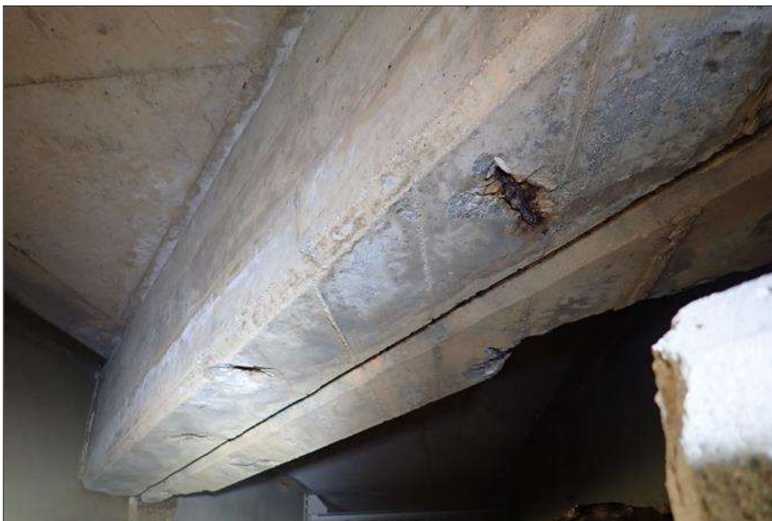
Span 2 Deck: bent 1 end diaphragm, bay 8, underside, (4) spalls (up to 7" diameter x 1") with exposed rusted rebar
