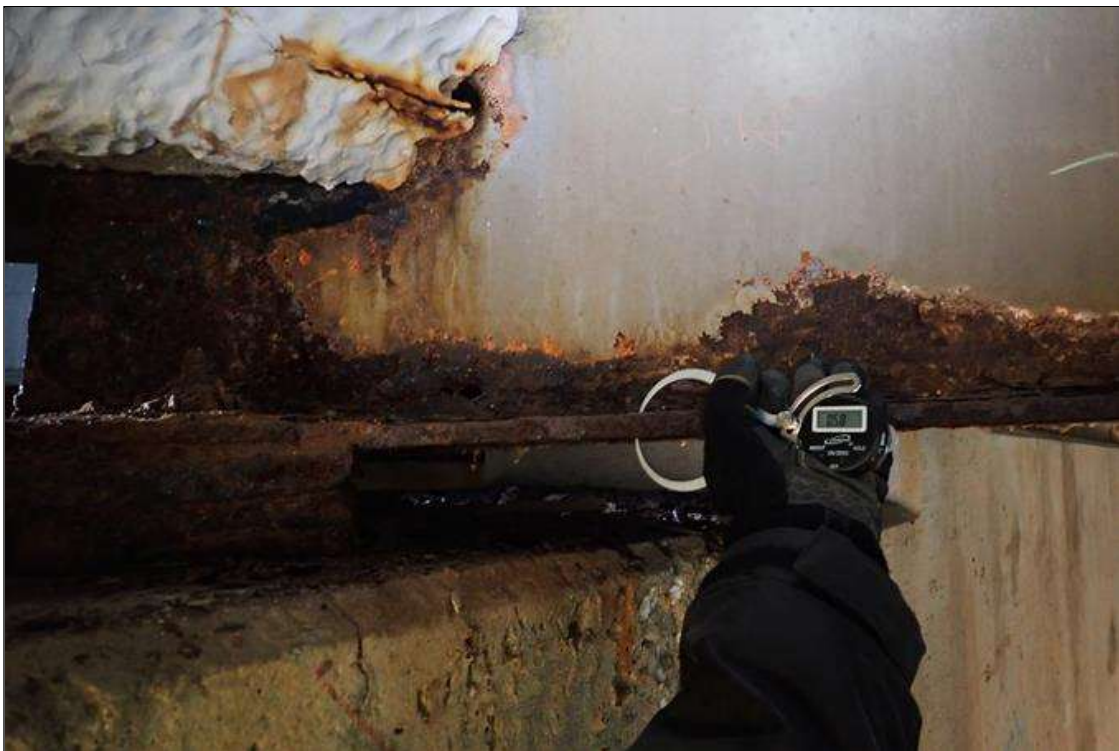
Span 2 Beam 7: (PAR) at bent 1, corrosion with section loss: bottom flange, (0.6" average remaining x 3'); web at bearing, (1/16" remaining x 1' x 16" high) with corrosion hole (2" x 1")
