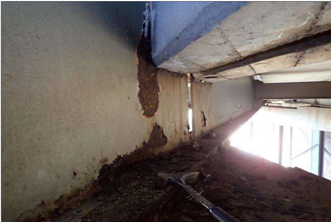
Span 5 Beam 10: at bent 4, corrosion with section loss: bottom of web and at end diaphragm, (1/16" loss x 2" x 1.5')
