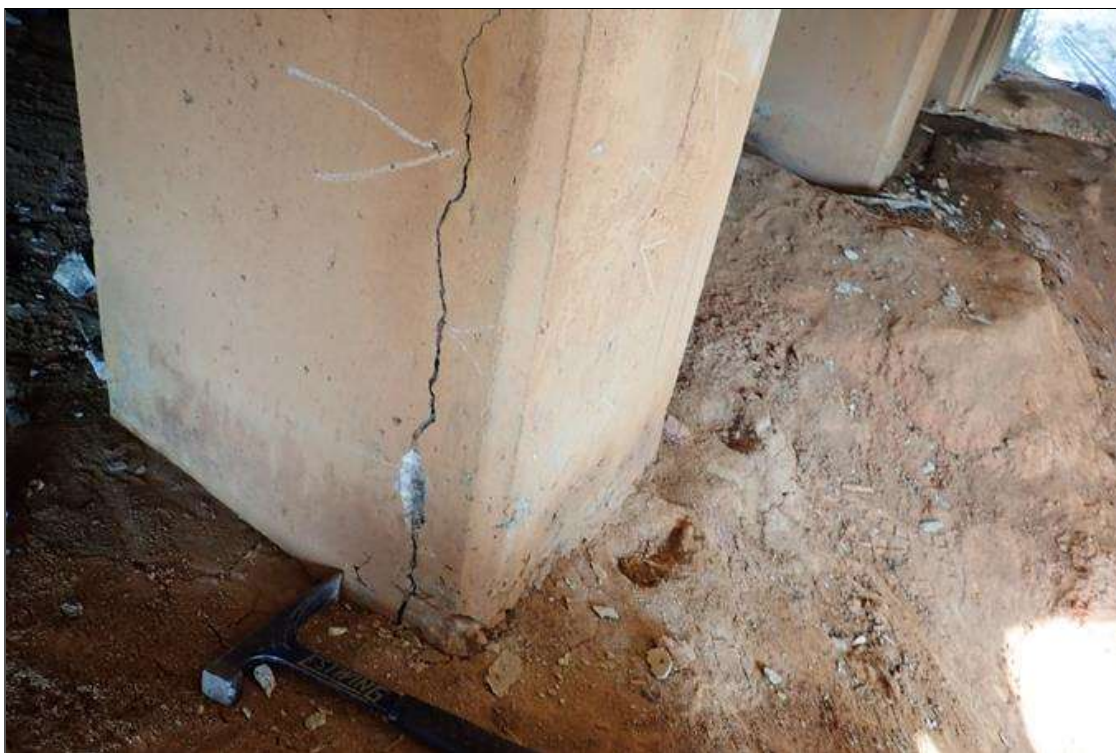
Bent 1 Pile 11: vertical cracks (up to 1/4" x 2')
