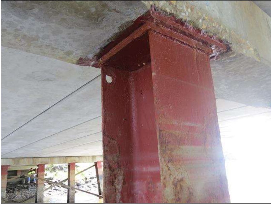
BENT 5 COLUMN 2 - 1/4IN TAPERED SECTION LOSS 1/4IN REMAINING AT NEAR RIGHT FLANGE EDGE. 1IN DIAMETER HOLE TOP OF FAR LEFT FLANGE. (PAR PHOTO)
