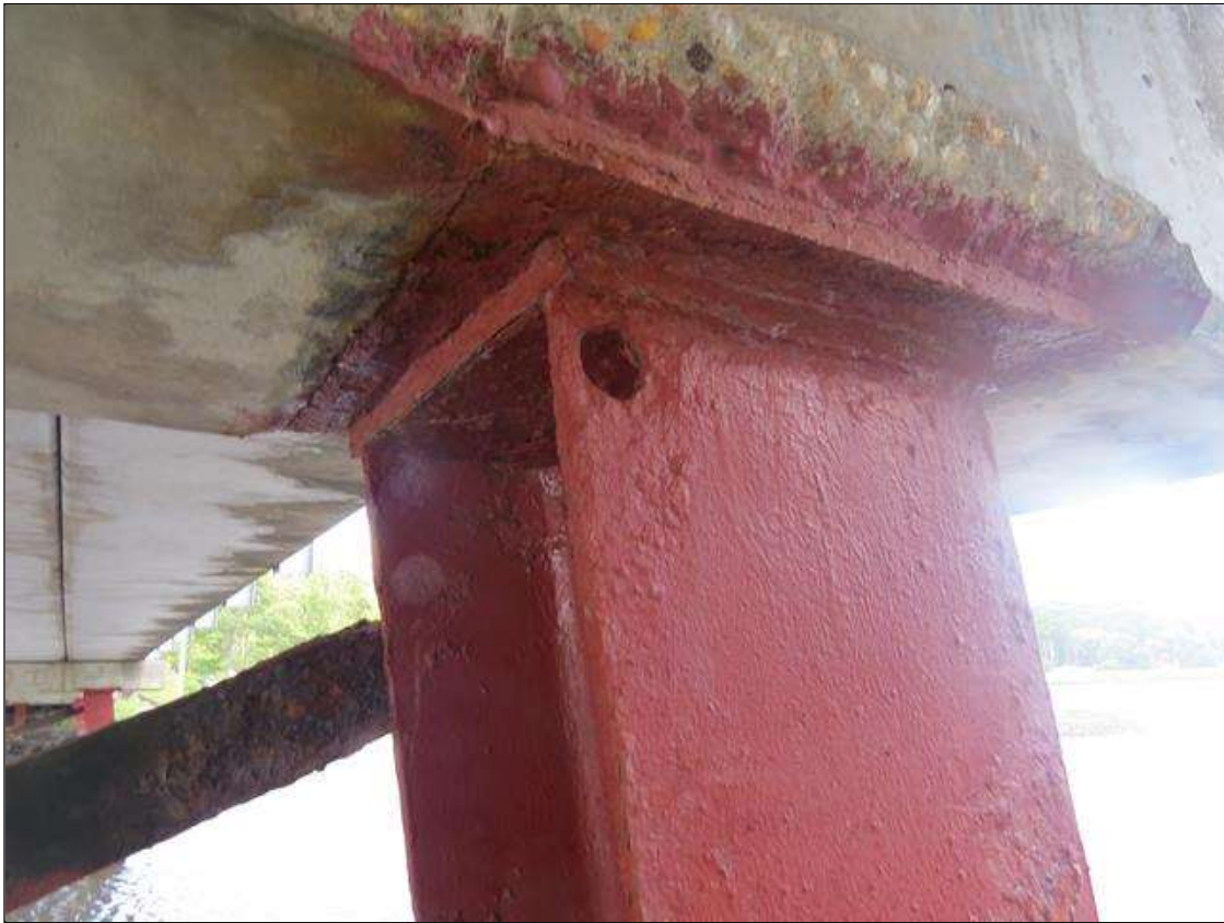
BENT 4 COLUMN 1 - 1/8IN TAPERED SECTION LOSS 3/8IN REMAINING AT ALL FLANGE EDGES
