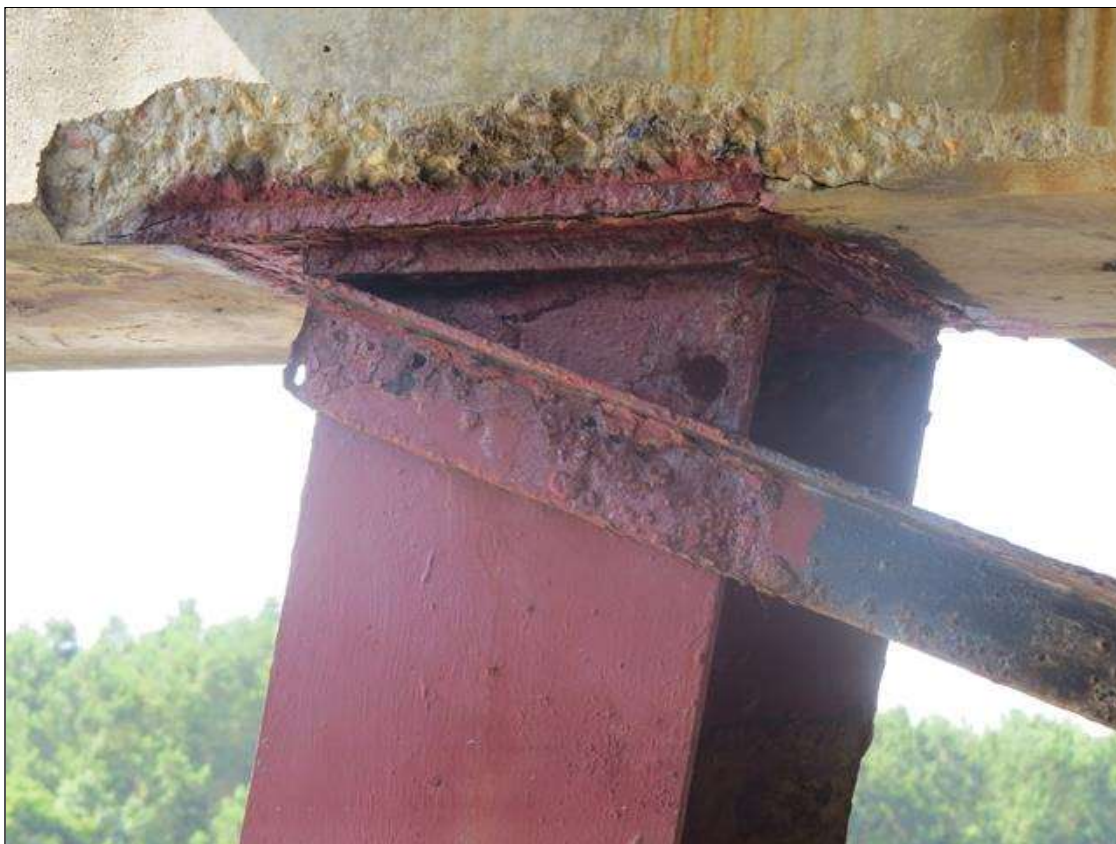
BENT 6 COLUMN 6 - KNIFE EDGING AT NEAR LEFT FLANGE. 1IN DIAMETER HOLE IN FAR LEFT FLANGE AT TOP. (PAR PHOTO)
