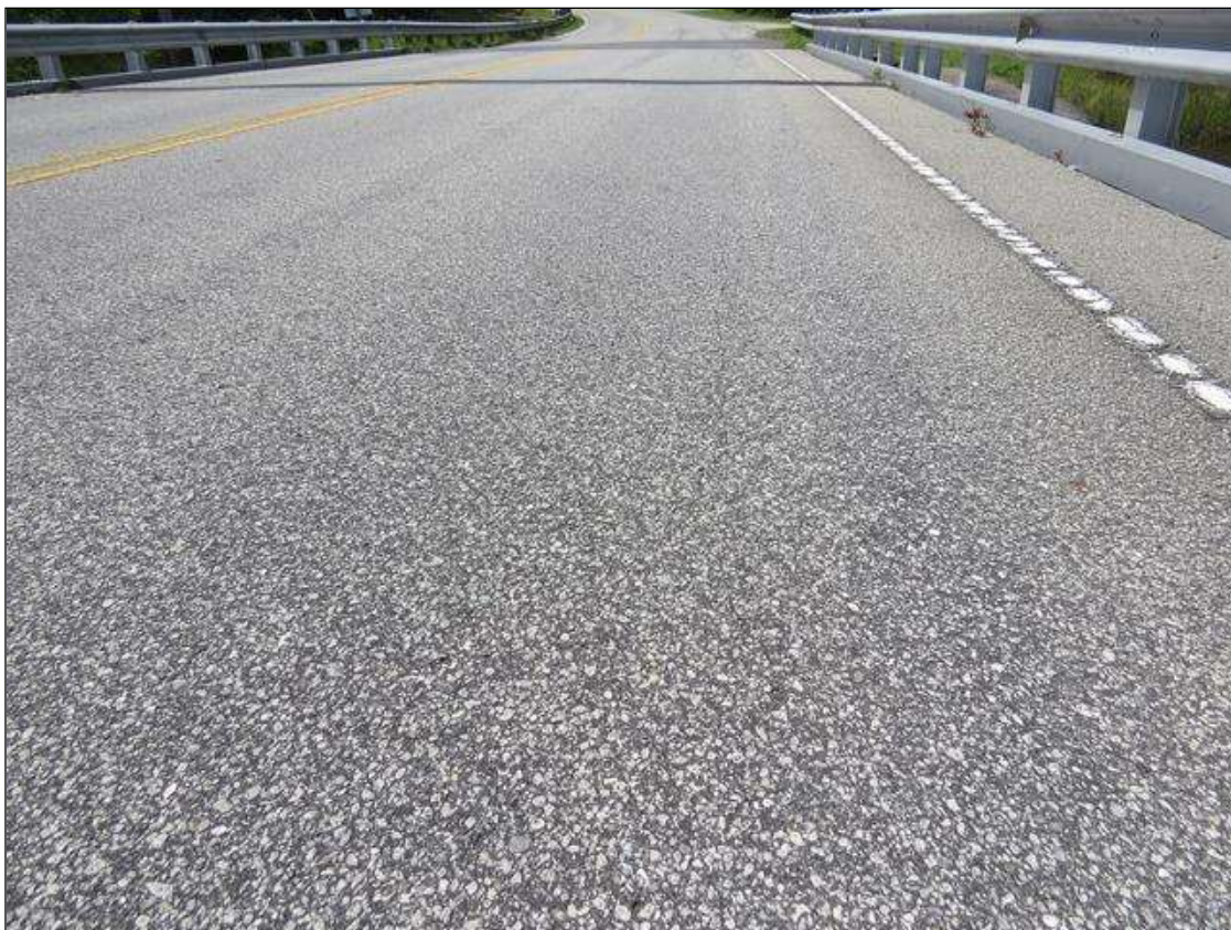
SPAN 6 AWS - HALF LENGTH HAIRLINE CRACK IN FAR HALF OF SPAN
