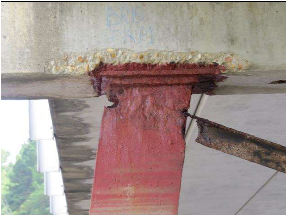
TYPICAL 100% DETERIORATION OF LATERAL BRACING, BENT 2 COLUMN 1 (PAR PHOTO)
