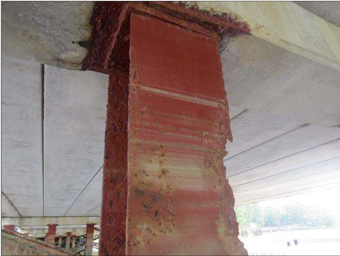
BENT 3 COLUMN 2 - 100% SECTION LOSS (2IN W X 12IN H) TO FAR LEFT FLANGE. 1/4IN TAPERED SECTION LOSS 1/4IN REMAINING AT ALL OTHER FLANGE EDGES 2FT FROM TOP. WEB IS HEAVILY PITTED. (PAR PHOTO)
