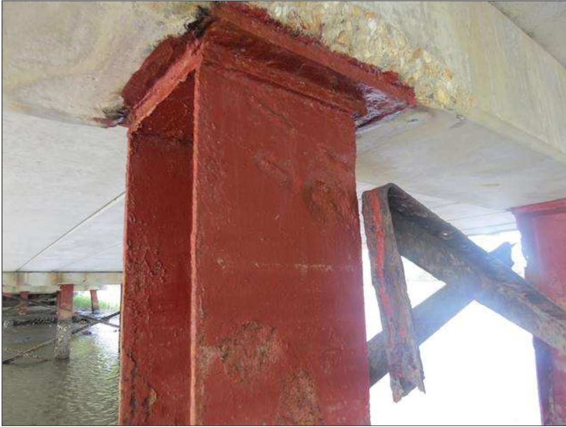
BENT 3 COLUMN 4 - 1/16IN TAPERED SECTION LOSS, 7/16IN REMAINING AT ALL FLANGE EDGES 2FT FROM TOP. TYPICAL 100% DETERIORATION OF LATERAL BRACING. (PAR PHOTO)
