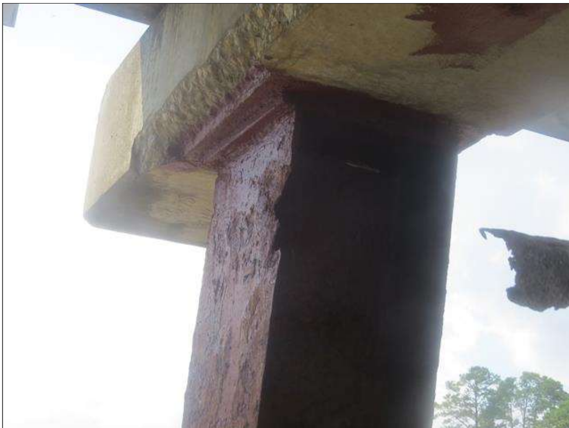
BENT 2 COLUMN 6 - 100% SECTION LOSS (2IN W X 6IN H) AT FAR LEFT FLANGE EDGE. 1/8IN TAPERED SECTION LOSS AT OTHER FLANGE EDGES. (PAR PHOTO)
