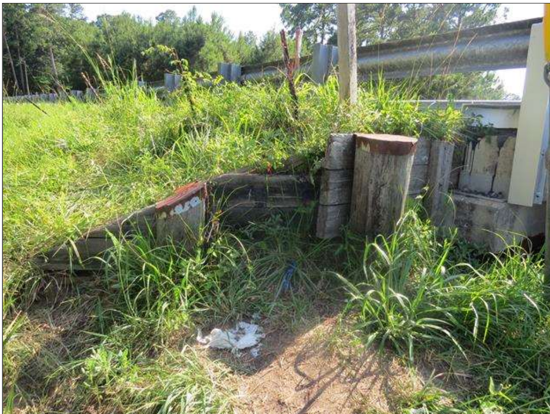
FAR LEFT WINGWALL, MODERTE DETERIORATION TO HORIZONTAL TIMBER LAGGING.
