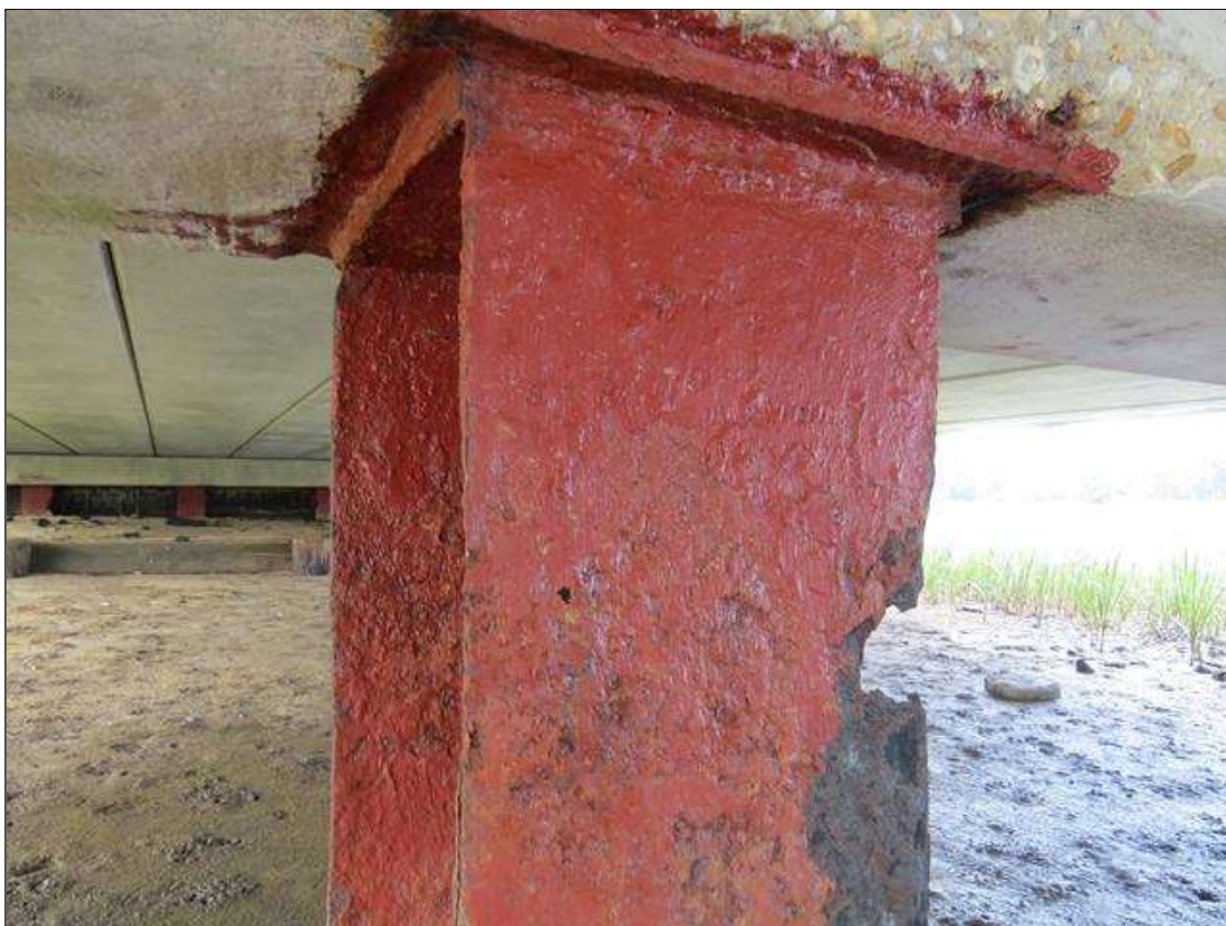
BENT 1 COLUMN 4 - 100% TAPERED SECTION LOSS (2IN W X 3 IN L) AT FAR LEFT FLANGE, 1/4IN TAPERED SECTION LOSS 1/4IN REMAINING AT OTHER FLANGES. (PAR PHOTO)
