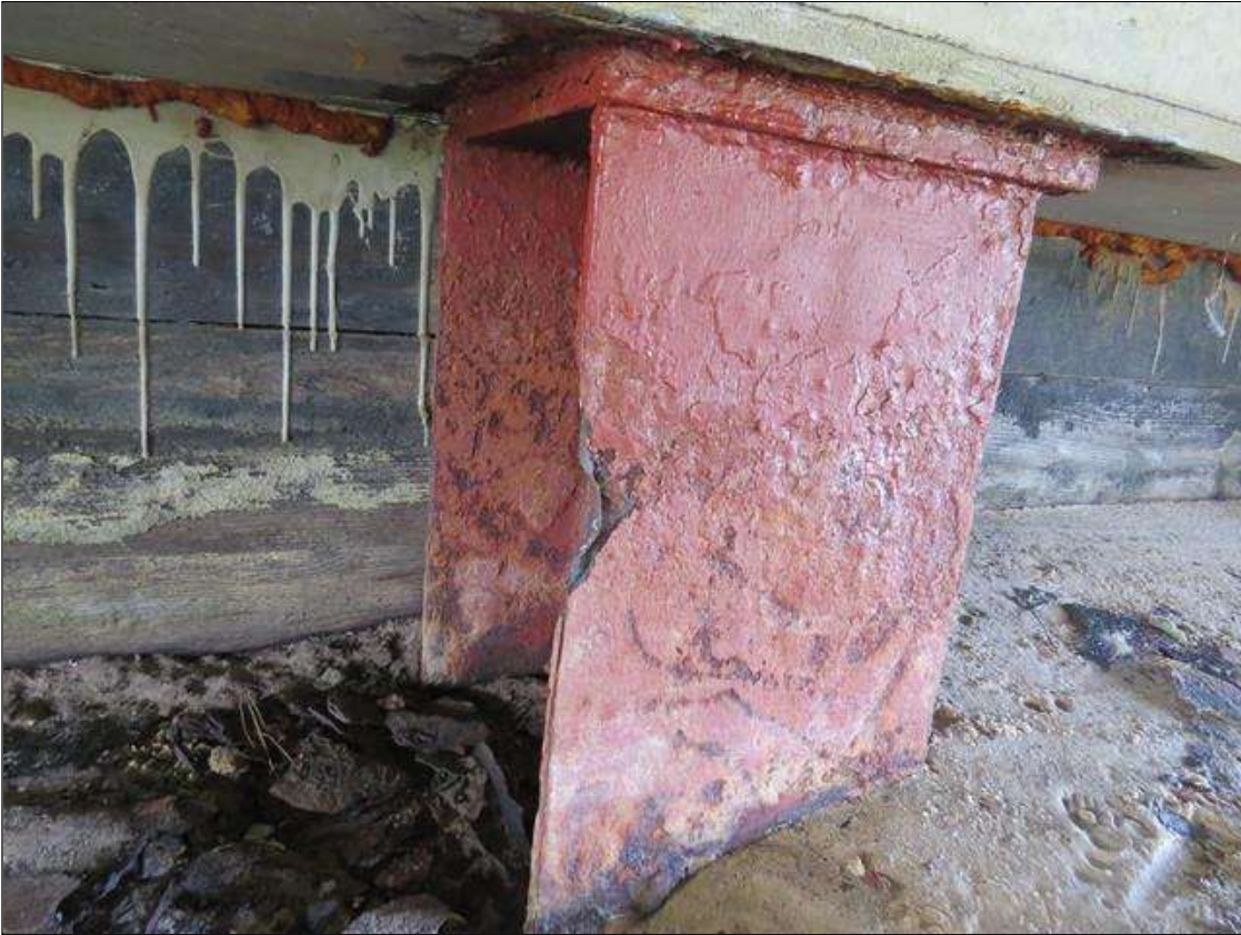
END BENT 1 COLUMN 3 - KNIFE EDGING TO FAR RIGHT FLANGE EDGE. 1/8IN TAPERED SECTION LOSS 3/8IN REMAINING TO REMAINING FLANGE EDGES. (PAR PHOTO)
