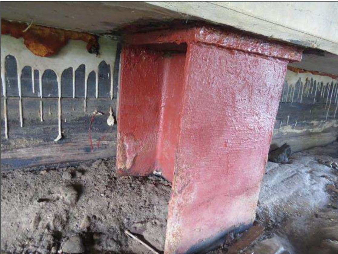
END BENT 1 COLUMN 4 - HEAVY SCALING TO FLANGE EDGES WITH NO MEASURABLE SECTION LOSS
