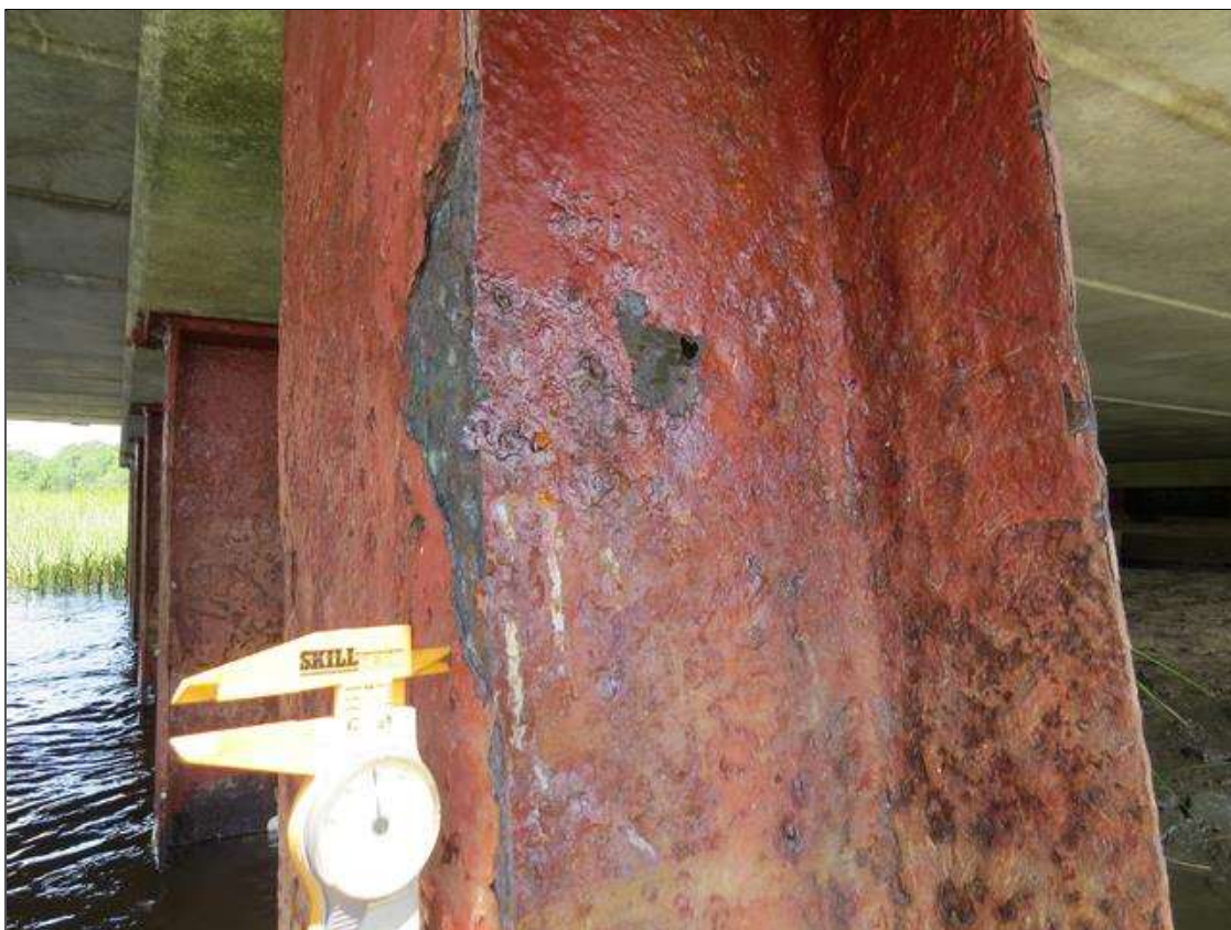
BENT 1 COLUMN 1 - KNIFE EDGING TO FAR FLANGES EDGES (UP TO 50% SECTION LOSS), 1/8IN TAPERED SECTION LOSS 3/8IN REMAINING TO NEAR FLANGES. (PAR PHOTO)
