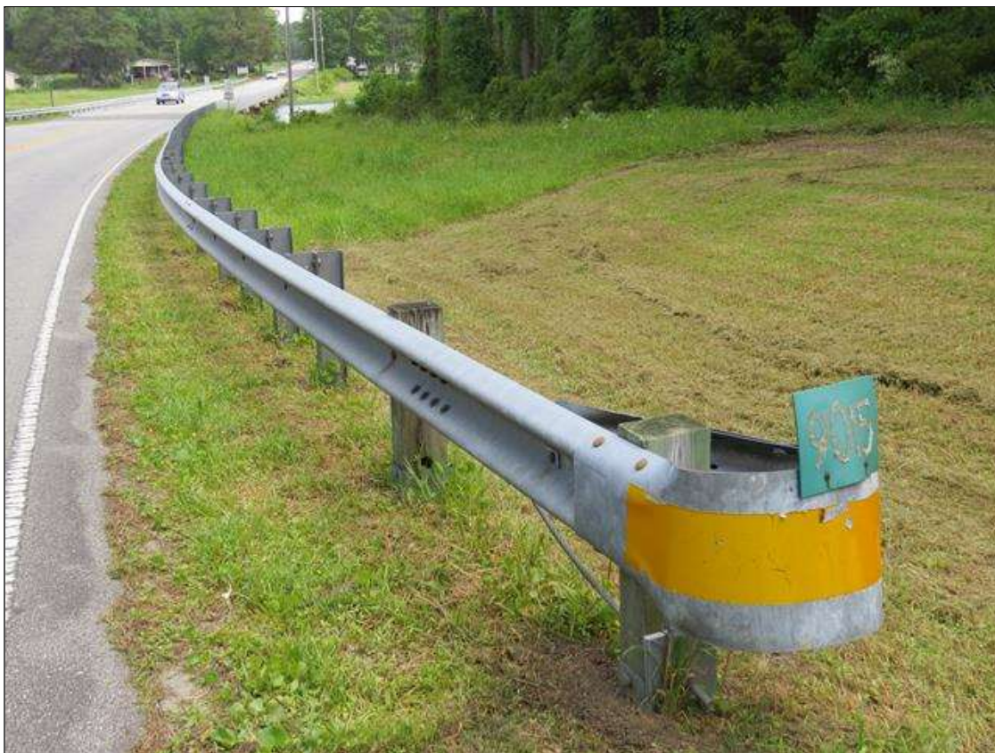
TYPICAL DELINEATOR END TREATMENT, MINOR COLLISION DAMAGE AT FAR LEFT
