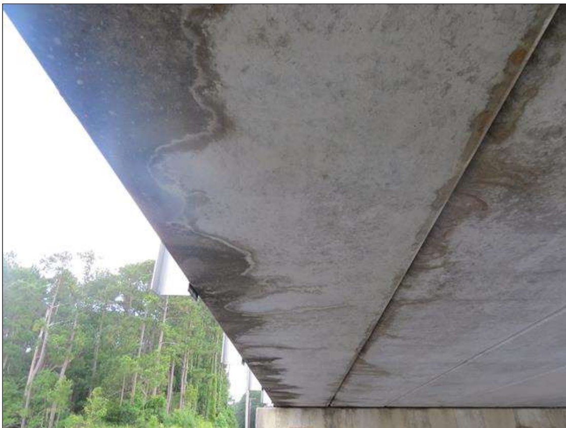
TYPICAL WATER STAINING TO LEFT FASCIA BEAM, SPAN 4 LOOKING AHEAD
