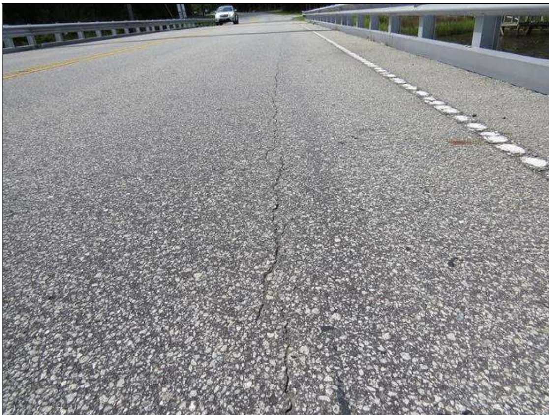
SPAN 5 AWS - FULL LENGTH OPEN LONGITUDINAL CRACK (1/4IN), 2.5FT FROM RIGHT LINE
