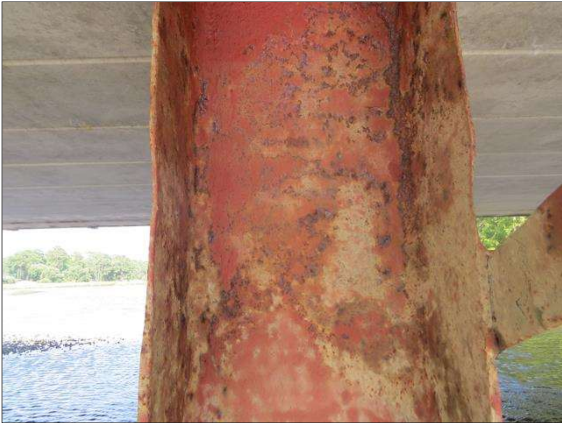
BENT 5 COLUMN 5 - KNIFE EDGING AT FAR RIGHT FLANGE WITH UP TO 50% SECTION LOSS. 3/8IN TAPERED SECTION LOSS 1/8IN REMAINING AT NEAR RIGHT. 1/4IN TAPERED SECTION LOSS 1/4IN REMAINING AT NEAR LEFT FLANGE EDGES. (PAR PHOTO)
