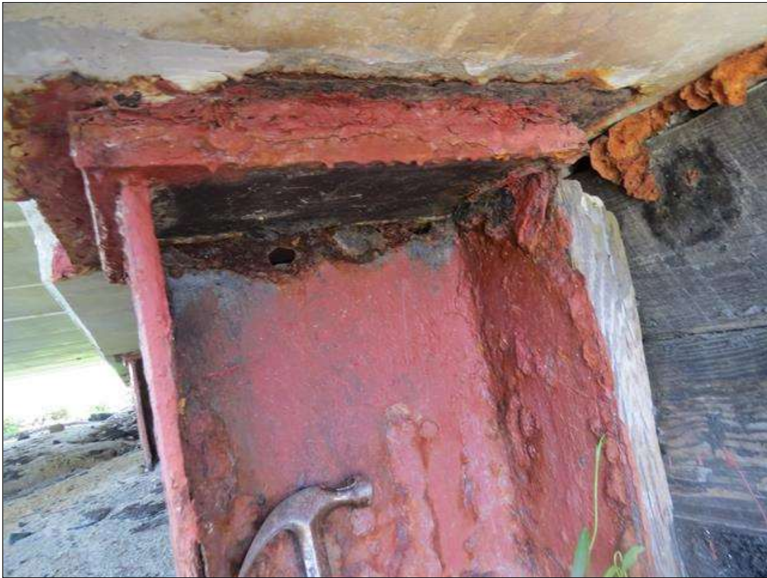
END BENT 1 COLUMN 1 - 1/8IN TAPERED SECTION LOSS 3/8IN REMAINING TO FLANGE EDGES. 50% SECTION LOSS TO TOP OF WEB. (PAR PHOTO)
