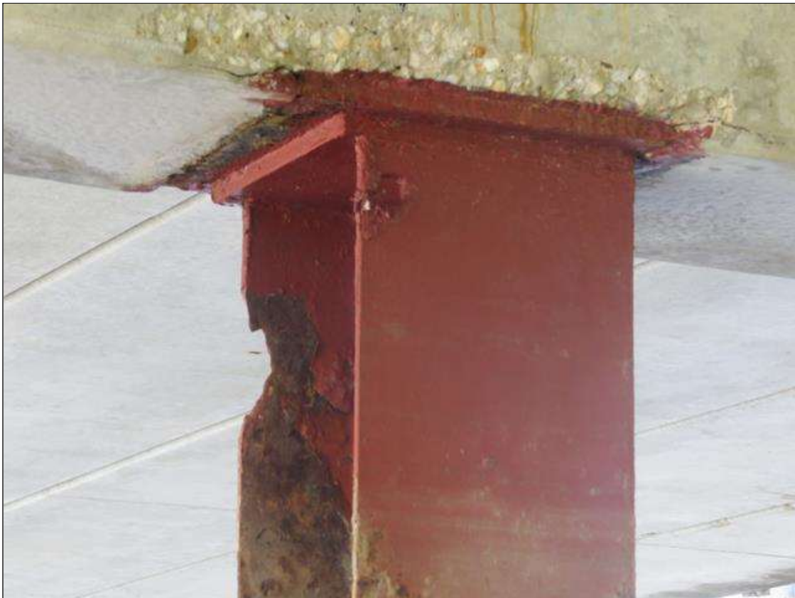
BENT 6 COLUMN 3 - 100% SECTION LOSS (2IN W X 6IN H) TO NEAR RIGHT FLANGE 1FT FROM TOP. 1/4IN TAPERED SECTION LOSS 1/4IN REMAINING AT ALL FLANGE EDGES 2FT FROM TOP. (PAR PHOTO)
