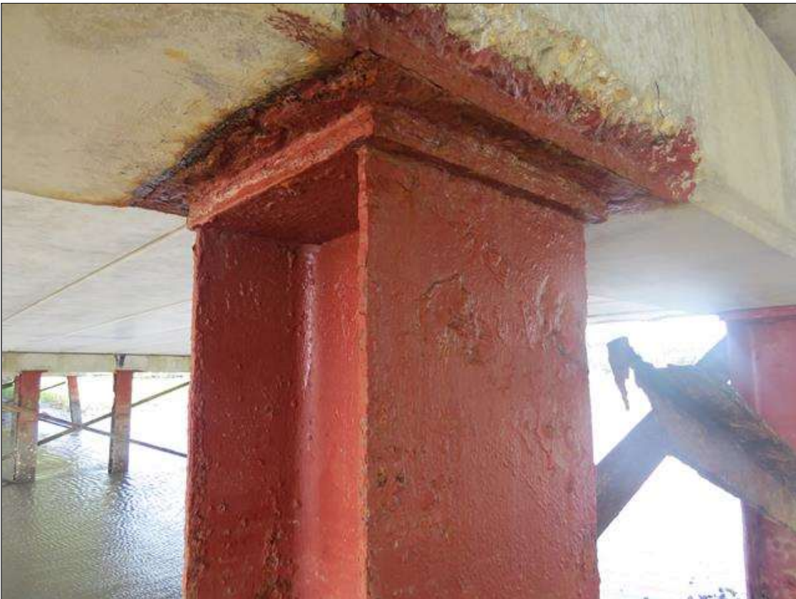
BENT 4 COLUMN 4 - 3/8IN TAPERED SECTION LOSS 1/8IN REMAINING AT FAR RIGHT FLANGE EDGE. 1/4IN TAPERED SECTION LOSS AT OTHER FLANGE EDGES. (PAR PHOTO)
