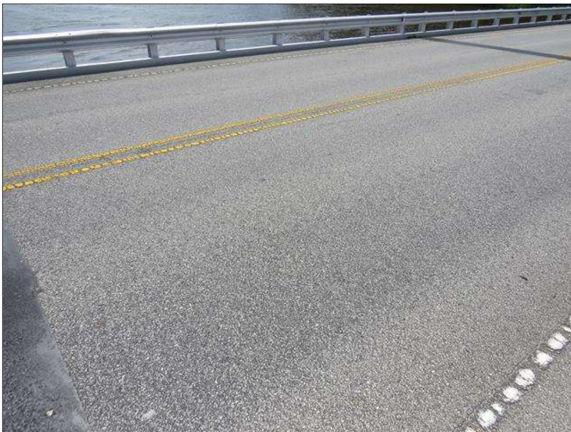
TYPICAL AWS, MODERATE TO HEAVY WEAR THROUGHOUT, SPAN 2
