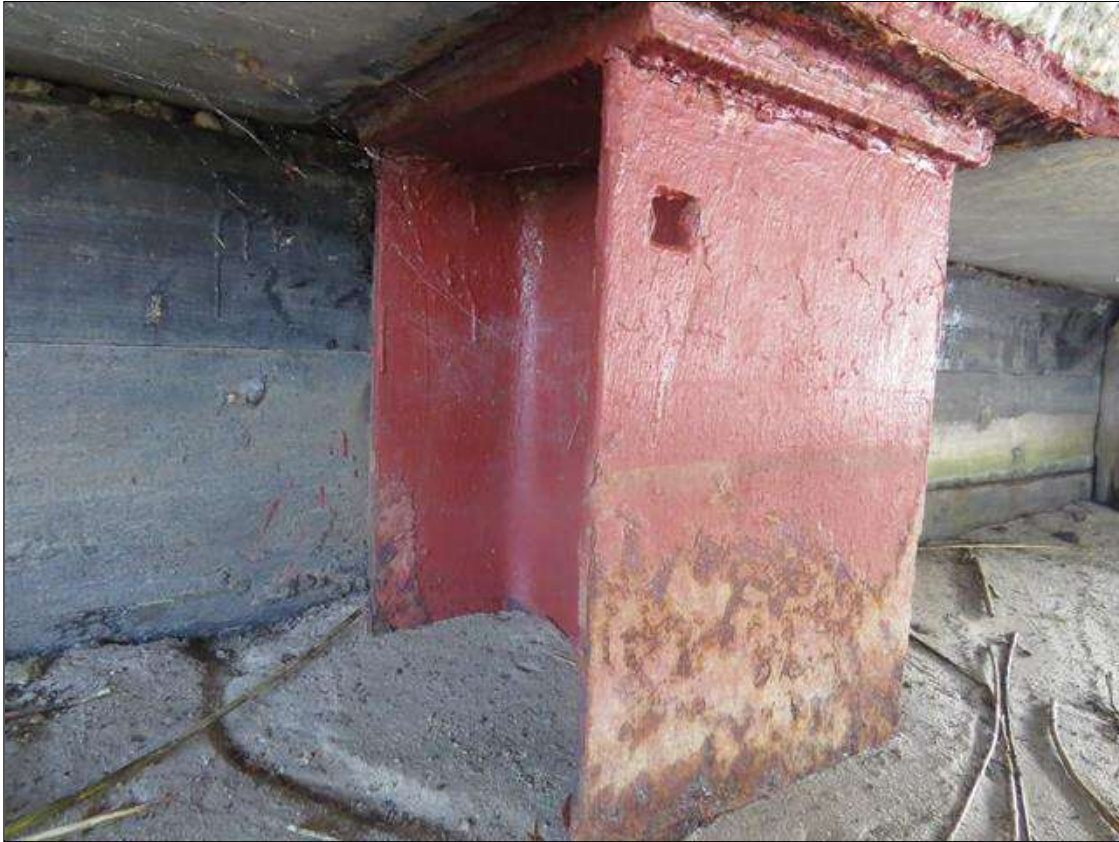
END BENT 2 COLUMN 2 - 1/4IN TAPERED SECTION LOSS 1/4IN REMAINING AT ALL FLANGE EDGES. 1IN X 1IN HOLE IN NEAR LEFT FLANGE AT TOP. (PAR PHOTO)
