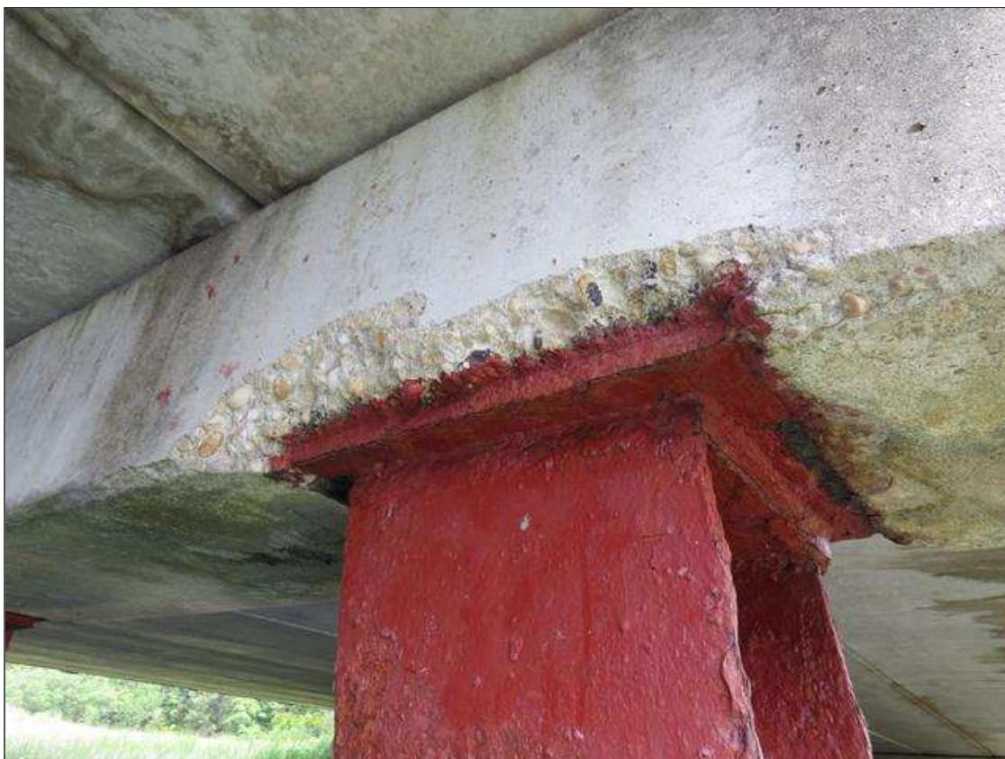
TYPICAL SPALLING ( UP TO 24IN X 3IN X 2IN) TO BOTH SIDES OF ALL CAPS AT ALL INTERIOR BENTS, BENT 1 COLUMN 1 FAR SIDE SHOWN
