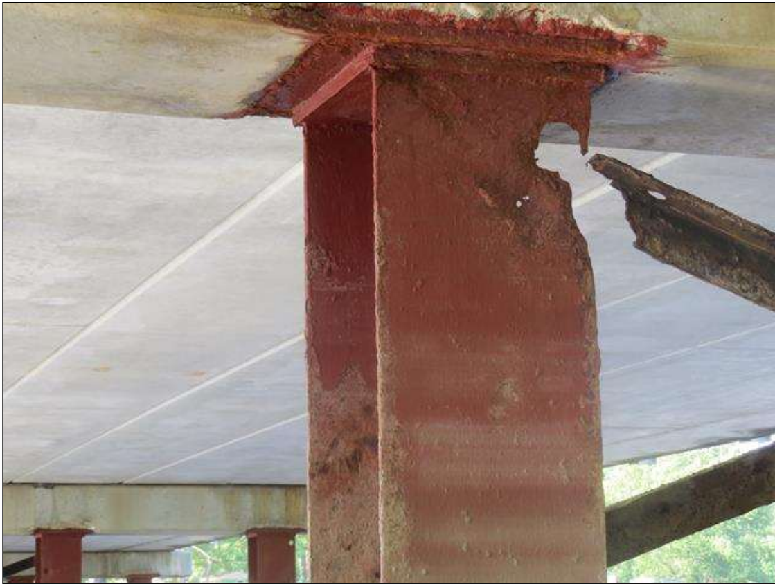
BENT 6 COLUMN 4 - 100% SECTION LOSS TO FAR LEFT FLANGE AT TOP. 1/4IN TAPERED SECTION LOSS 1/4IN REMAINING AT ALL FLANGE EDGES 2-FT FROM TOP. (PAR PHOTO)
