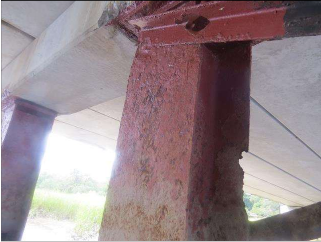
BENT 2 COLUMN 4 - KNIFE EDGING WITH 100% SECTION LOSS (1INW X 8IN H) AT FAR RIGHT FLANGE. 1/4IN TAPERED SECTION LOSS 1/4IN REMAINING AT FAR RIGHT, 1/8IN TAPERED SECTION LOSS AT NEAR RIGHT. (PAR PHOTO)
