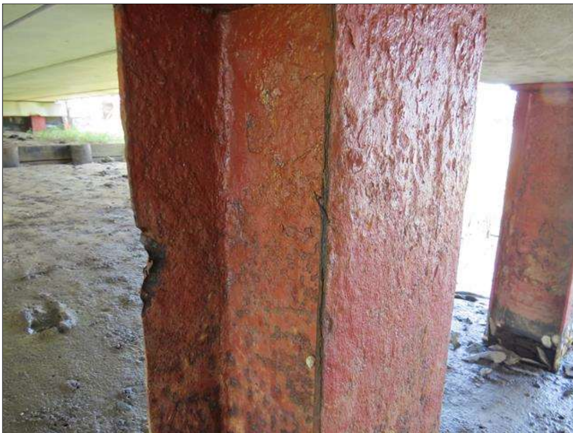
BENT 1 COLUMN 3 - KNIFE EDGING TO NEAR RIGHT FLANGE. 1/8IN TAPERED SECTION LOSS 3/8IN REMAINING AT OTHER FLANGES. (PAR PHOTO)
