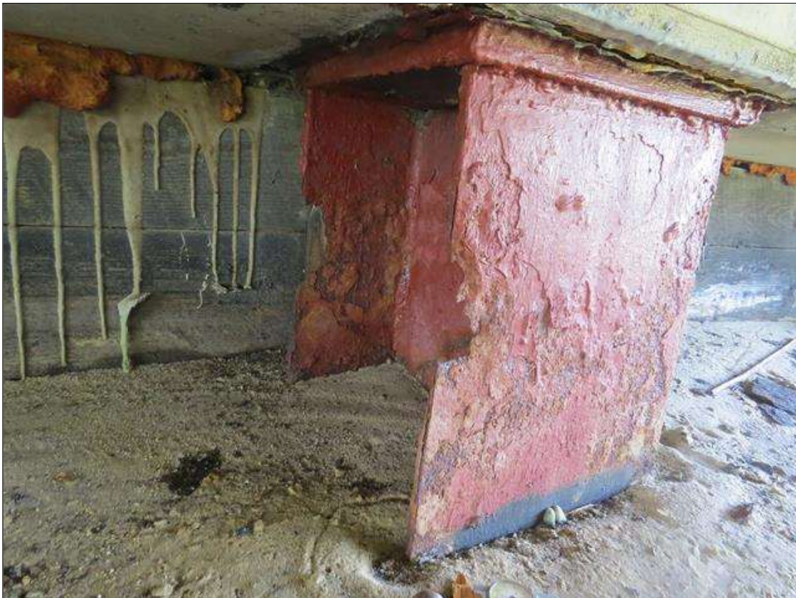
END BENT 1 COLUMN 2 - 100% SECTION LOSS TO RIGHT FLANGE EDGES (UP TO 6IN H X 2IN W) 1/8IN TAPERED SECTION LOSS 3/8IN REMAINING TO LEFT FLANGE EDGES. (PAR PHOTO)
