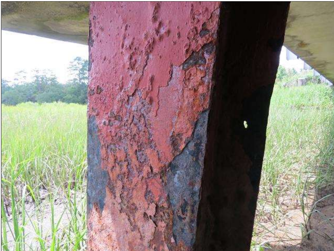
BENT 1 COLUMN 6 - KNIFE EDGING ON LEFT FLANGE EDGES. 1/4IN SECTION LOSS 1/4IN REMAINING AT FAR RIGHT. 1/8IN TAPERED SECTION LOSS 3/8IN REMAINING AT NEAR RIGHT. (PAR PHOTO)
