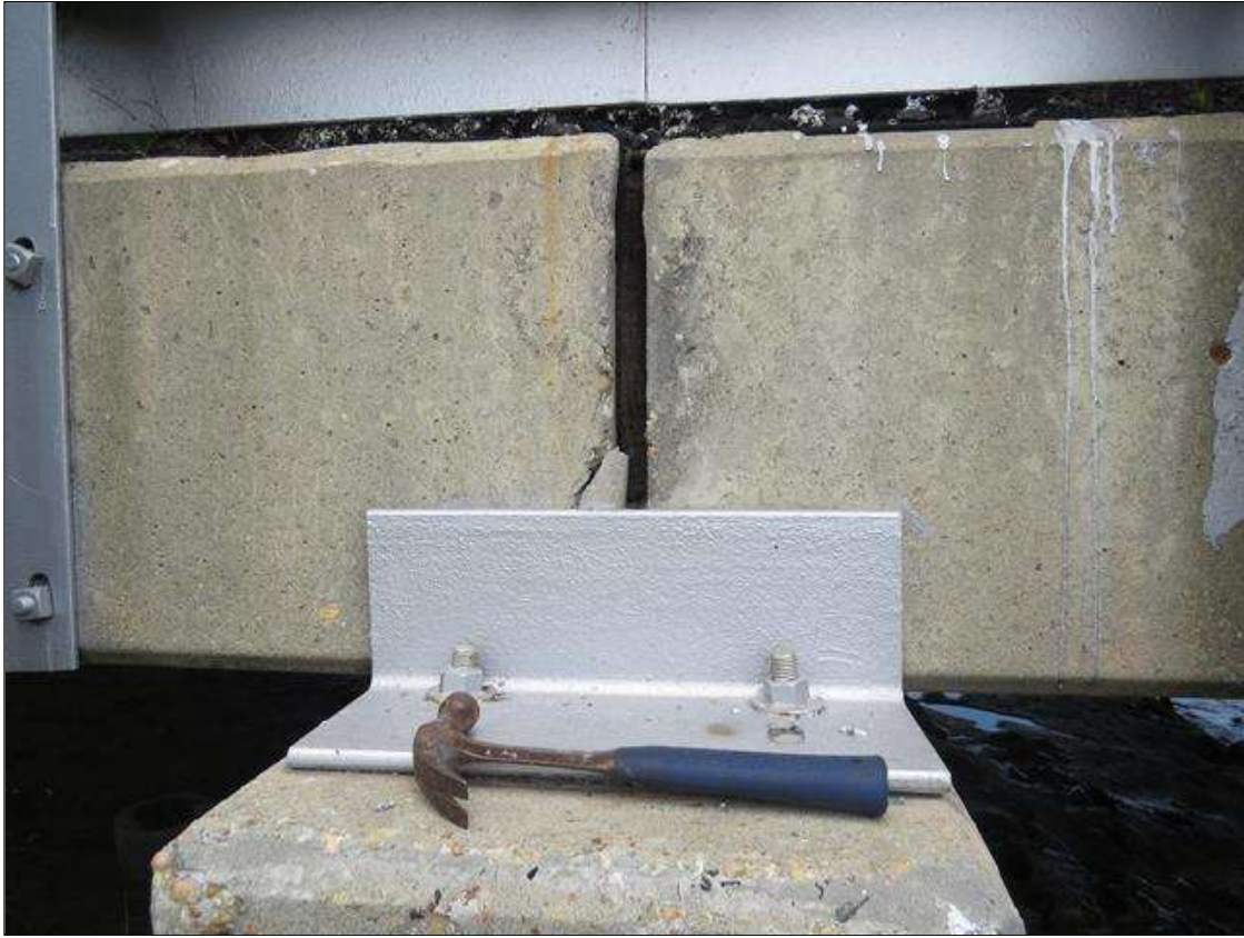
SPAN 1 BEAM 11 - SPALL (9IN H X 3IN W) AT FAR END ON RIGHT SIDE
