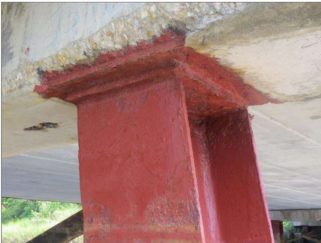
BENT 5 COLUMN 6 - HEAVY PITTING WITH UP TO 50% SECTION LOSS TO NEAR RIGHT AND FAR RIGHT FLANGES. (PAR PHOTO)
