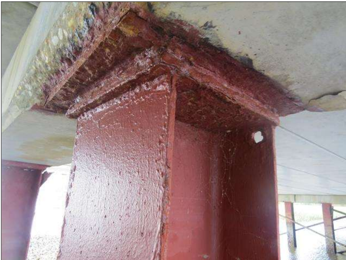
BENT 4 COLUMN 2 - 1/16IN TAPERED SECTION LOSS 7/16IN REMAINING AT ALL FLANGE EDGES. 1IN DIAMETER HOLE IN NEAR LEFT FLANGE.
