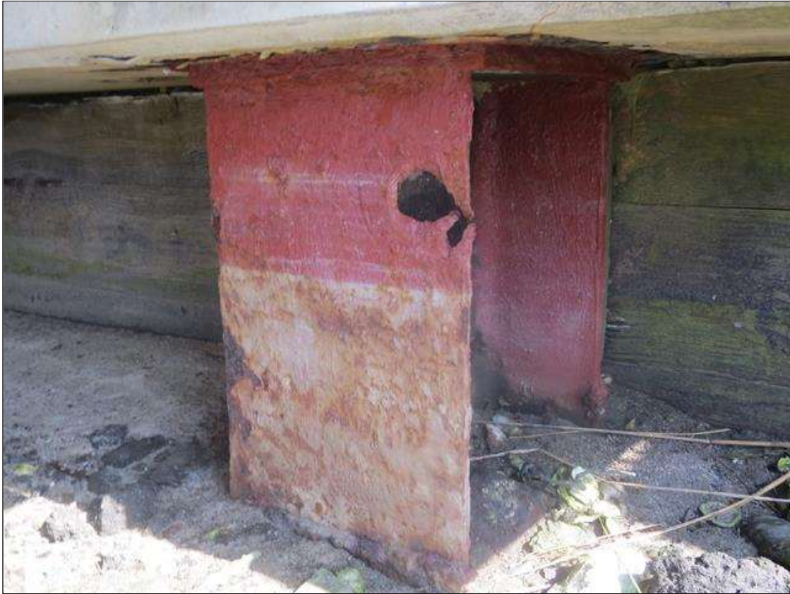
END BENT 2 COLUMN 6 - 100% SECTION LOSS (3IN W X 2IN H) AT NEAR RIGHT FLANGE AT TOP. 1/4IN TAPERED SECTION LOSS 1/4IN REMAINING AT ALL FLANGE EDGES AT GROUND LINE. (PAR PHOTO)
