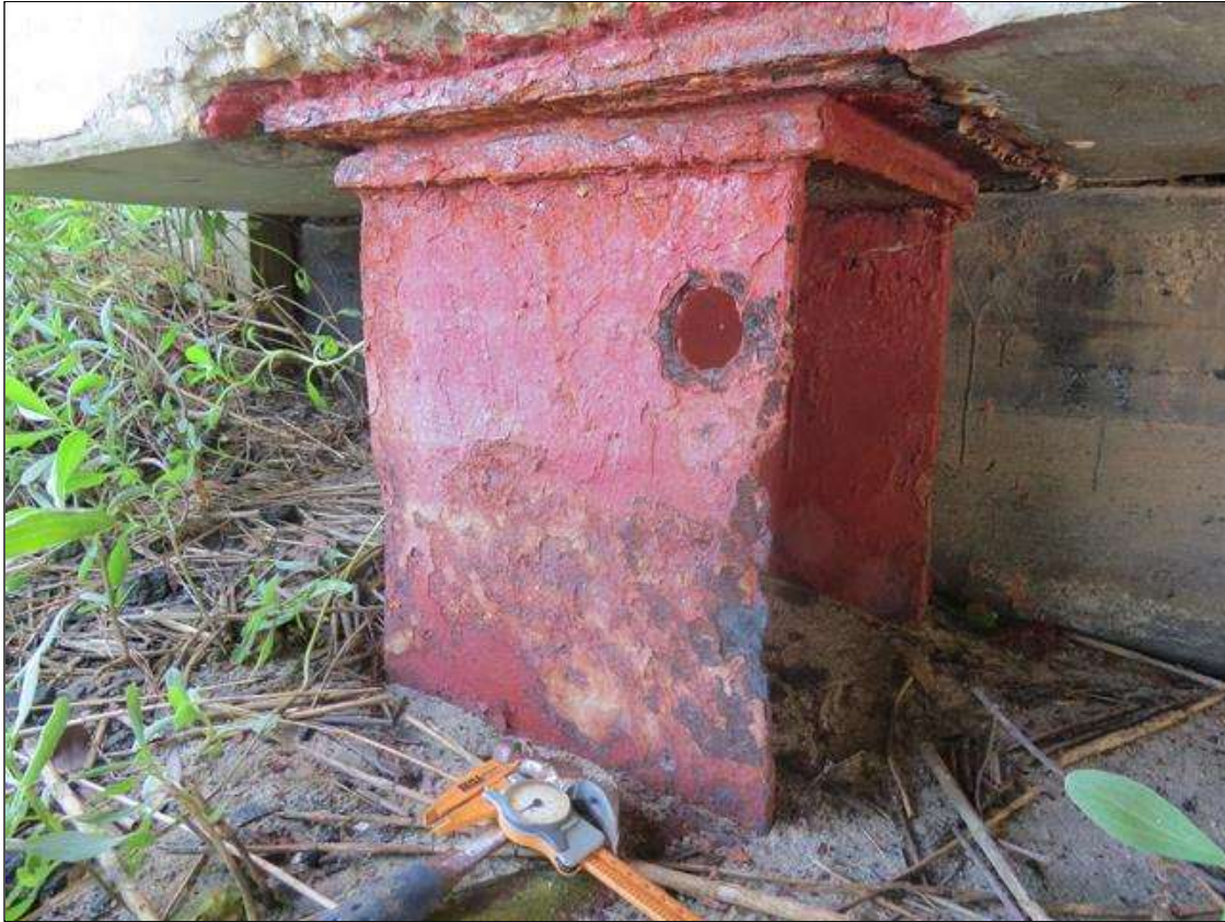
END BENT 2 COLUMN 1 - KNIFE EDGING WITH UP TO 50% SECTION LOSS TO THE NEAR RIGHT FLANGE. 1/4IN TAPERED SECTION LOSS 1/4IN REMAINING AT NEAR LEFT FLANGE EDGE. 1/16IN SECTION LOSS AT FAR FLANGE EDGES. (PAR PHOTO)
