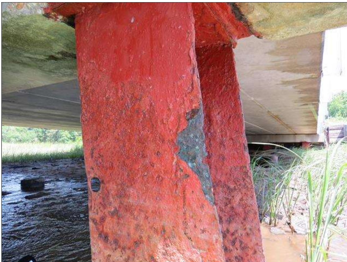
BENT 1 COLUMN 1 - KNIFE EDGING TO FAR FLANGES EDGES (50% SECTION LOSS), 1/8IN TAPERED SECTION LOSS 3/8IN REMAINING TO NEAR FLANGES. (PAR PHOTO)
