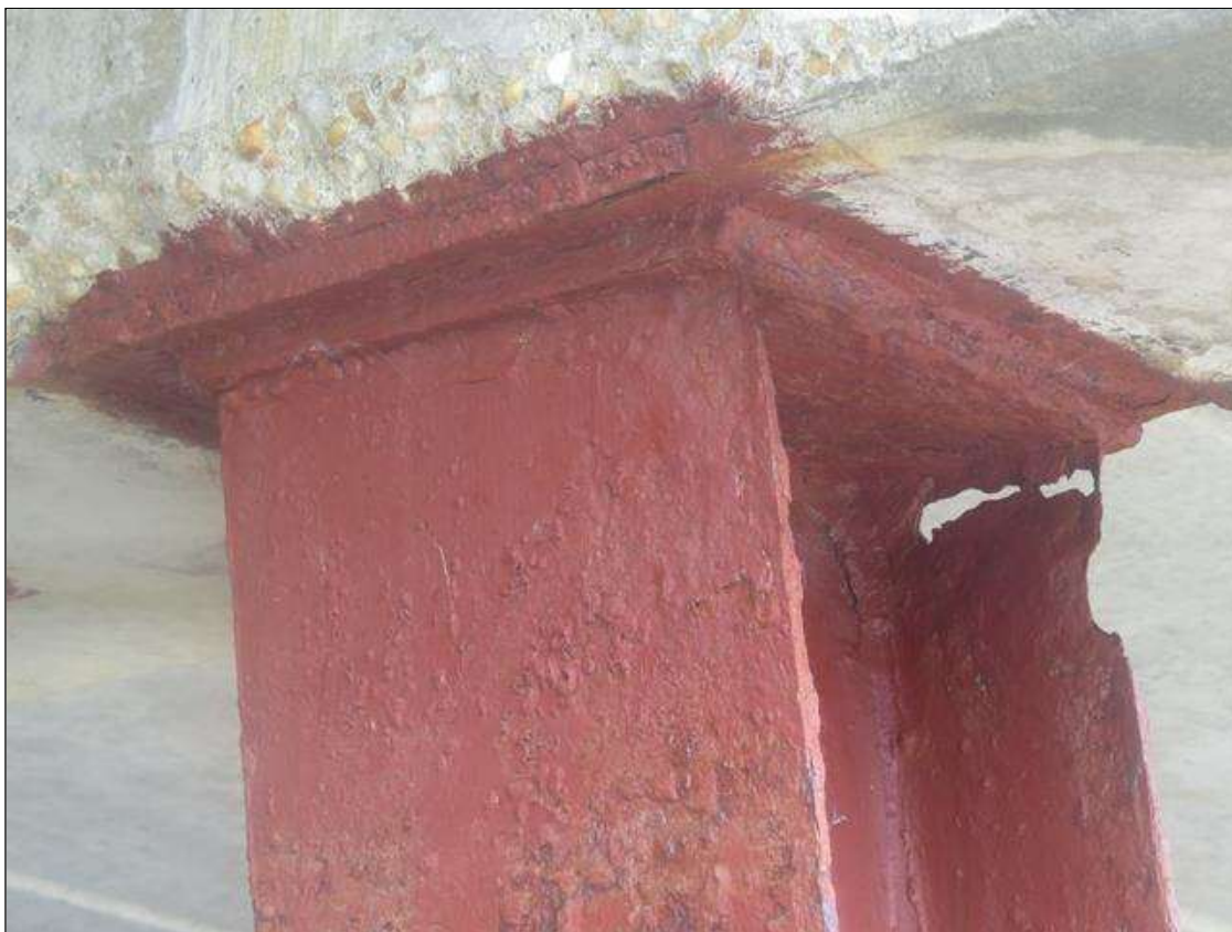
BENT 3 COLUMN 6 - 100% SECTION LOSS TO FAR RIGHT FLANGE AT TOP, 1/4IN TAPERED SECTION LOSS 1/4IN REMAINING ALL OTHER FLANGES. (PAR PHOTO)
