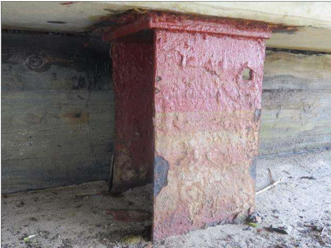
END BENT 2 COLUMN 5 - 3/8IN TAPERED SECTION LOSS 1/8IN REMAINING AT NEAR FLANGE EDGES AND FAR LEFT FLANGE EDGE. 1/4IN TAPERED SECTION LOSS AT FAR RIGHT. (PAR PHOTO)
