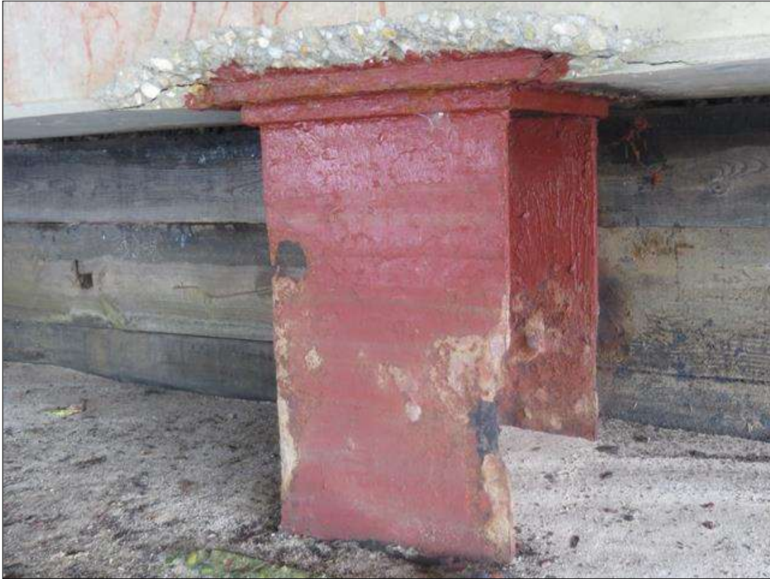
END BENT 2 COLUMN 4 - KNIFE EDGING TO NEAR RIGHT FLNGE WITH UP TO 50% SECTION LOSS. 1/4IN TAPERED SECTION LOSS 1/4IN REMAINING AT ALL FLANGE EDGES. (PAR PHOTO)
