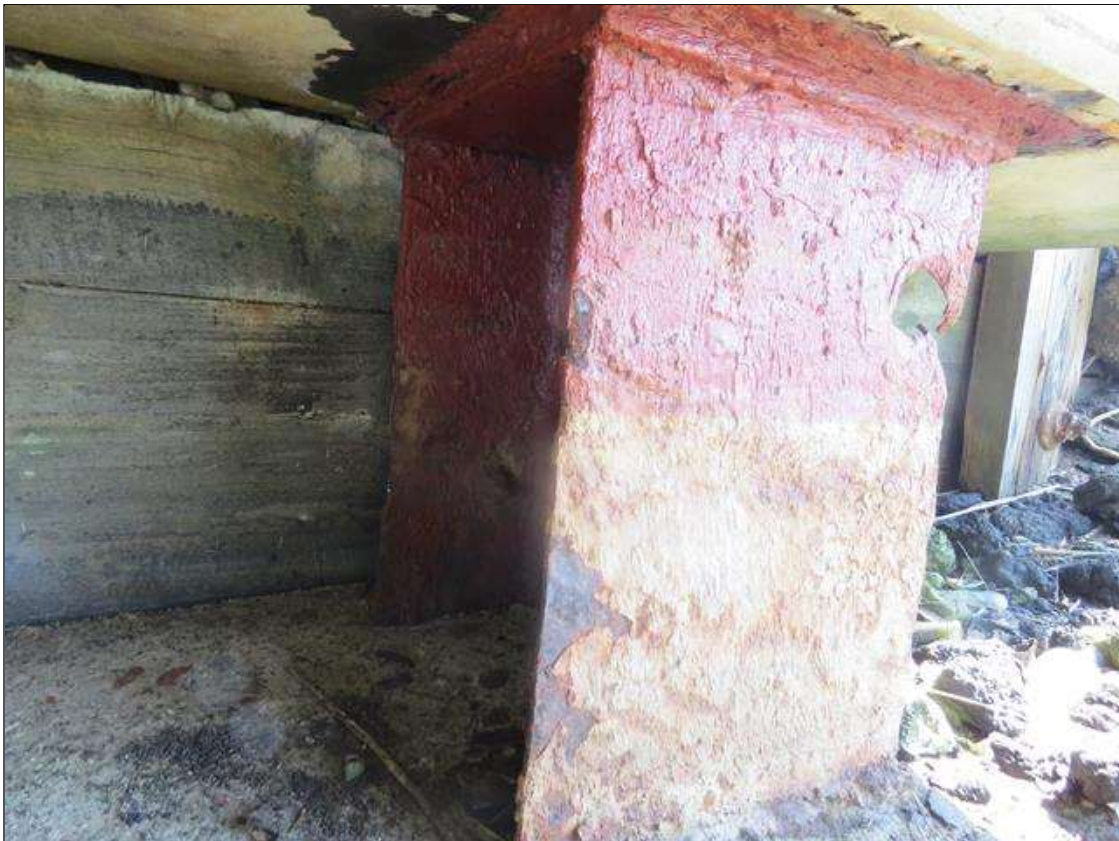
END BENT 2 COLUMN 3 - KNIFE EDGING WITH UP TO 50% SECTION LOSS TO NEAR LEFT AND FAR RIGHT FLANGES. 1/4IN TAPERED SECTION LOSS 1/4IN REMAINING AT ALL FLANGE EDGES. (PAR PHOTO)
