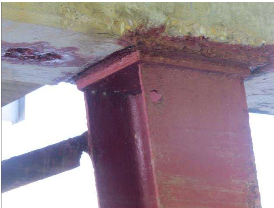
BENT 6 COLUMN 1 - 1/4IN TAPERED SECTION LOSS 1/4IN REMAINING AT ALL FLANGE EDGE 2FT FROM TOP. 1IN DIAMETER HOLE TOP OF FAR RIGHT FLANGE. (PAR PHOTO)
