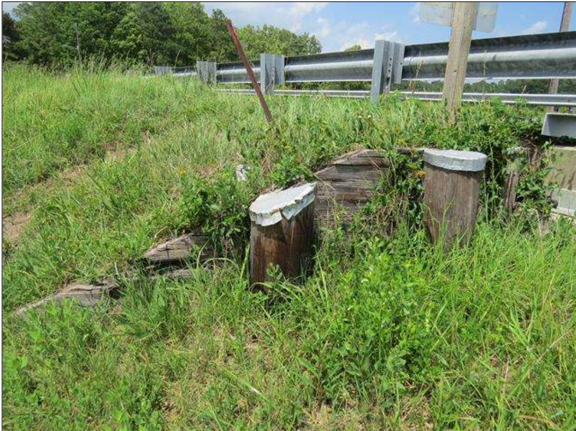
NEAR RIGHT WINGWALL - HEAVY DETERIORATION TO HORIZONTAL TIMBER LAGGING AT ENDS
