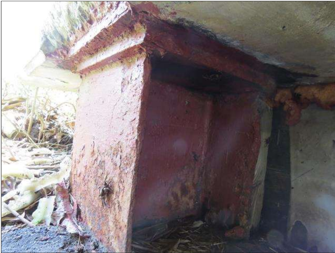
END BENT 1 COLUMN 6 - KNIFE EDGING TO NEAR LEFT FLANGE EDGE. 1/8IN TAPERED SECTION LOSS 3/8IN REMAINING TO OTHER FLANGE EDGES. (PAR PHOTO)
