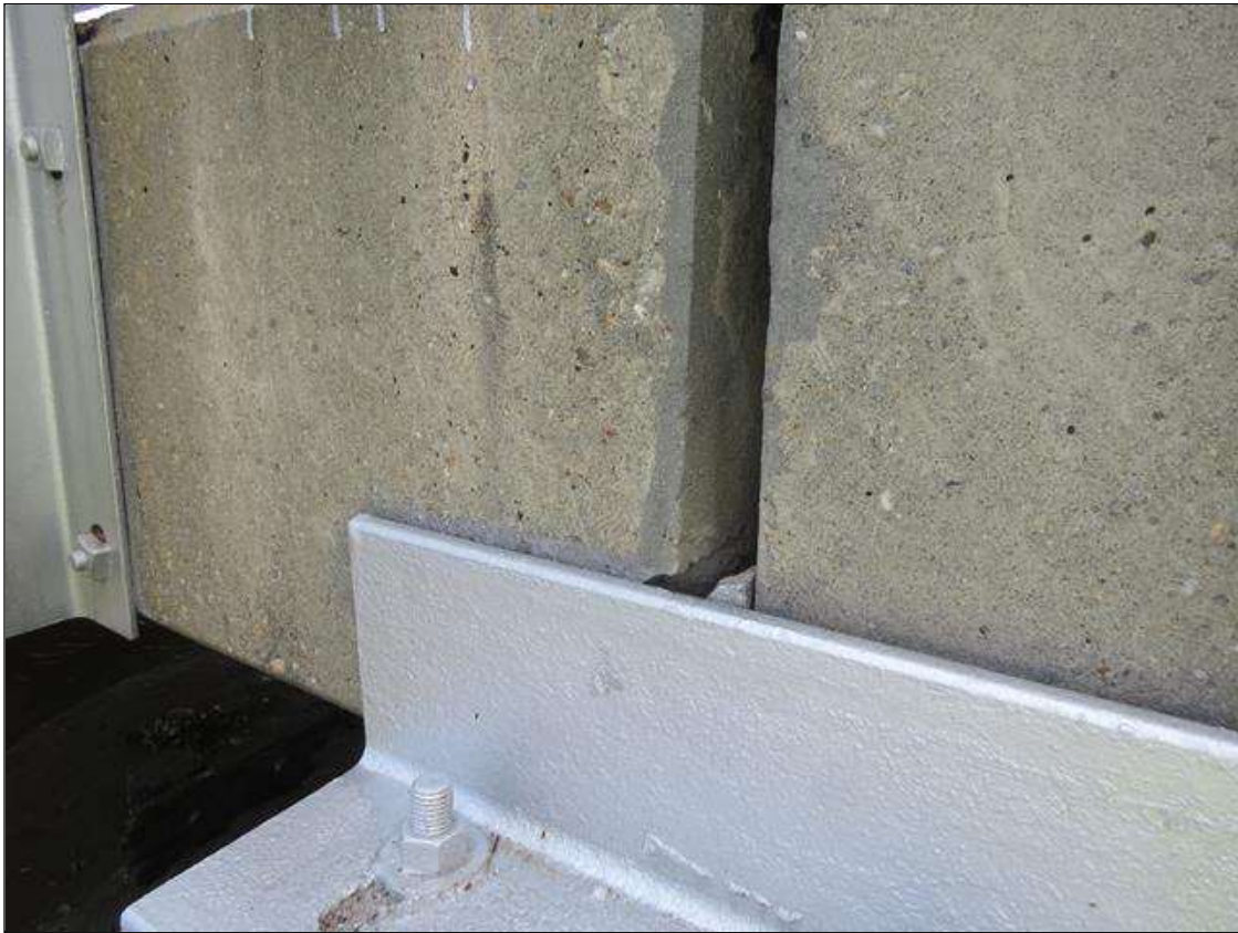
SPAN 2 BEAM 1 - SPALL (6IN H X 3IN W) AT NEAR LEFT END
