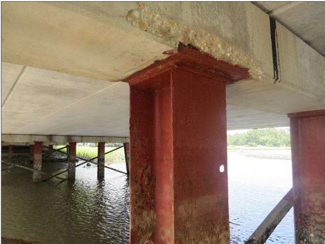
BENT 3 COLUMN 5 - 1/8IN TAPERED SECTION LOSS, 3/8IN REMAINING AT ALL FLANGE EDGES 2FT FROM TOP. 1IN DIAMETER HOLE IN FAR LEFT FLANGE.
