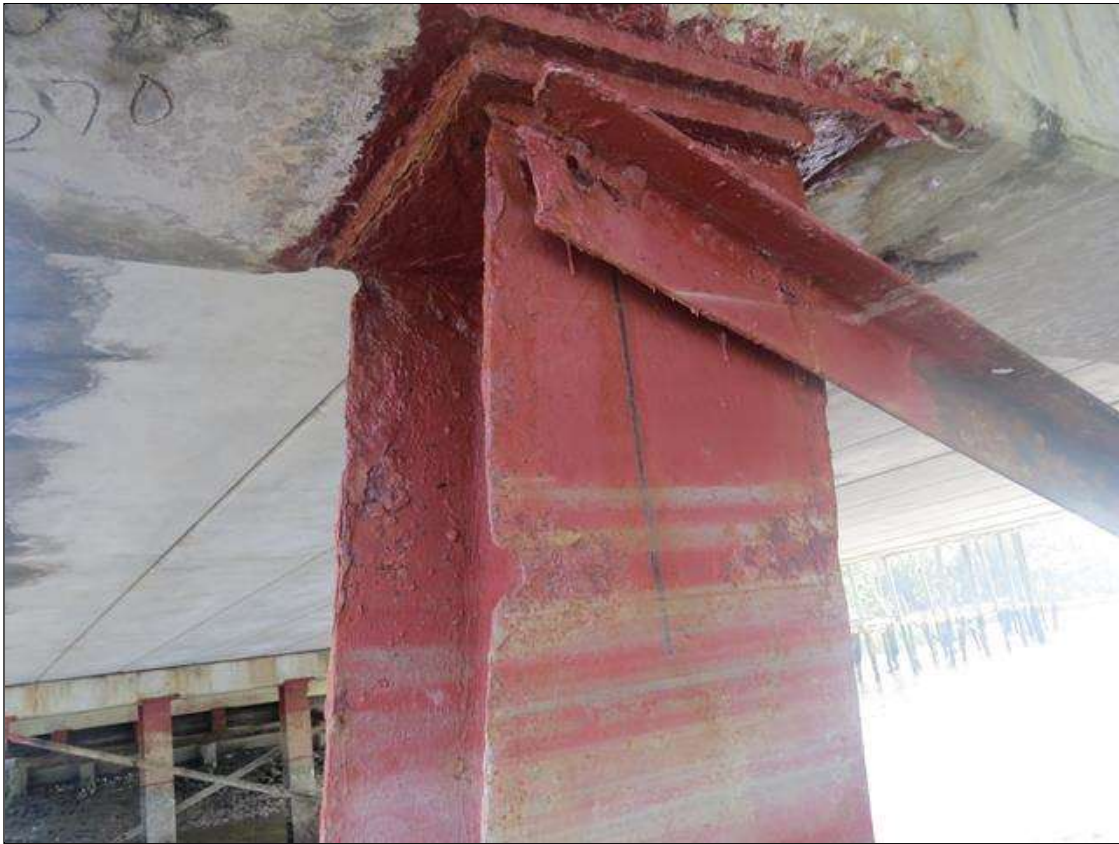
BENT 5 COLUMN 1 - KNIFE EDGING WITH UP TO 50% SECTION LOSS WITH A 1IN X 1IN SECTION OF 100% SECTION LOSS AT EDGE. 1/4IN TAPERED SECTION LOSS 1/4IN REMAINING AT OTHER FLANGE EDGES. (PAR PHOTO)
