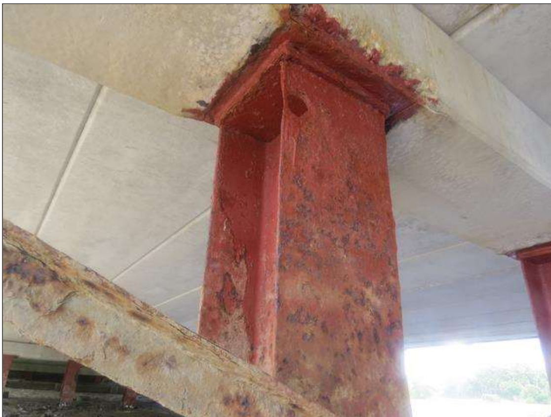
BENT 2 COLUMN 5 - 3/8IN TAPERED SECTION LOSS 1/8IN REMAINING AT FAR RIGHT, 3/8IN REMAINING OTHER FLANGE EDGES. (PAR PHOTO)
