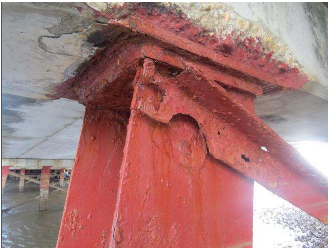
TYPICAL DETACHED LATERAL BRACING, BENT 4 AT COLUMN 2 (PAR PHOTO)
