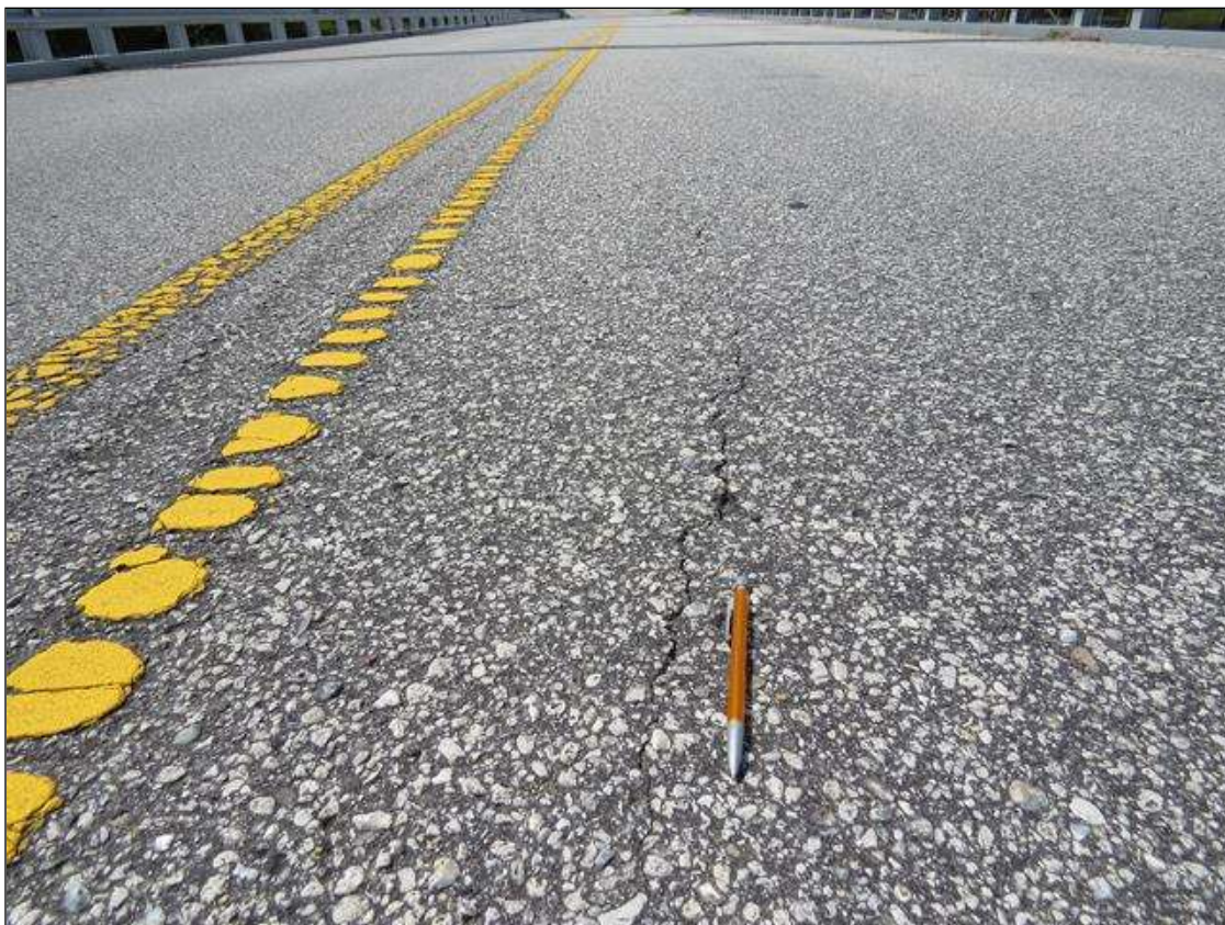
SPAN 2 AWS, OPEN LONGITUDINAL CRACK (1/8IN X 5FT) CENTER OF SPAN IN RIGHT LANE
