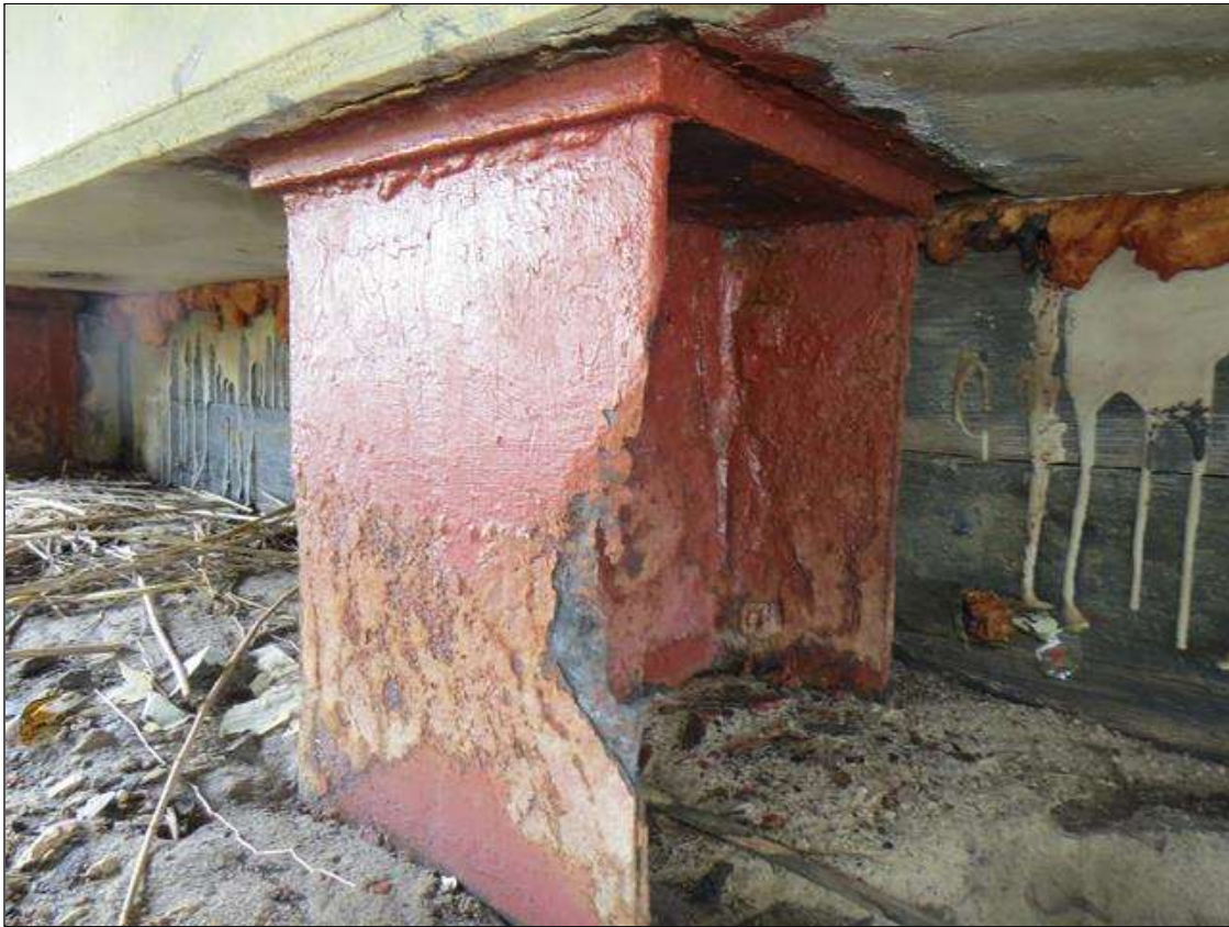
END BENT 1 COLUMN 5 - KNIFE EDGING WITH 100% SECTION LOSS (1IN W X 6IN H) AT FAR LEFT FLANGE. 3/8IN TAPERED SECTION LOSS 1/8IN REMAINING TO FAR RIGHT FLANGE EDGE. 1/8IN TAPERED SECTION LOSS 3/8IN REMAINING TO NEAR FLANGE EDGES. (PAR PHOTO)
