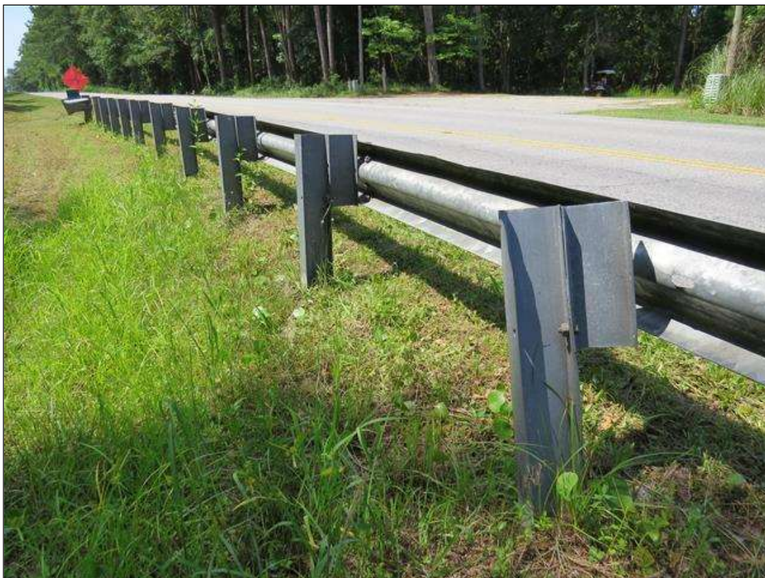
FAR LEFT APPROACH GUARDRAIL- DISCONNECTED & DAMAGED POST 50FT FROM END TREATMENT
