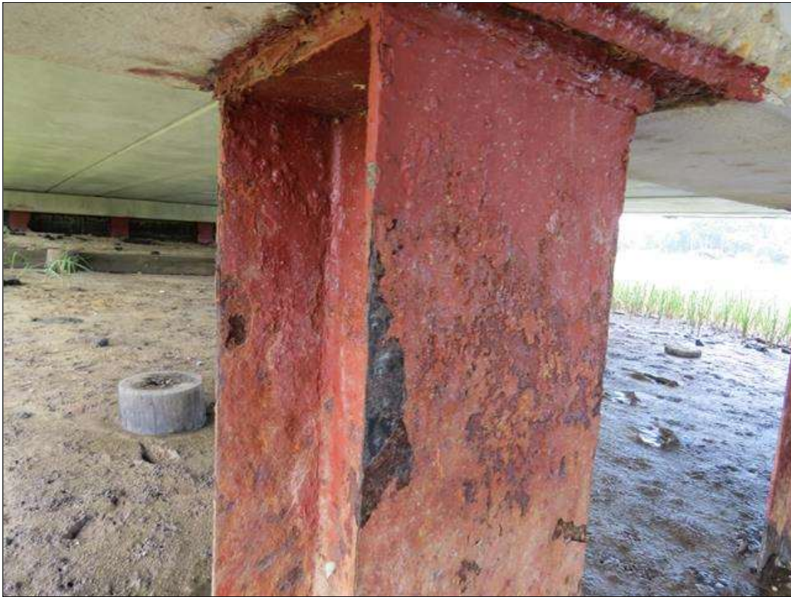
BENT 1 COLUMN 5 - 3/8IN SECTION LOSS 1/8IN REMAINING AT FAR RIGHT FLANGE, 1/4IN SECTION LOSS 1/4IN REMAINING AT OTHER FLANGE EDGES. (PAR PHOTO)
