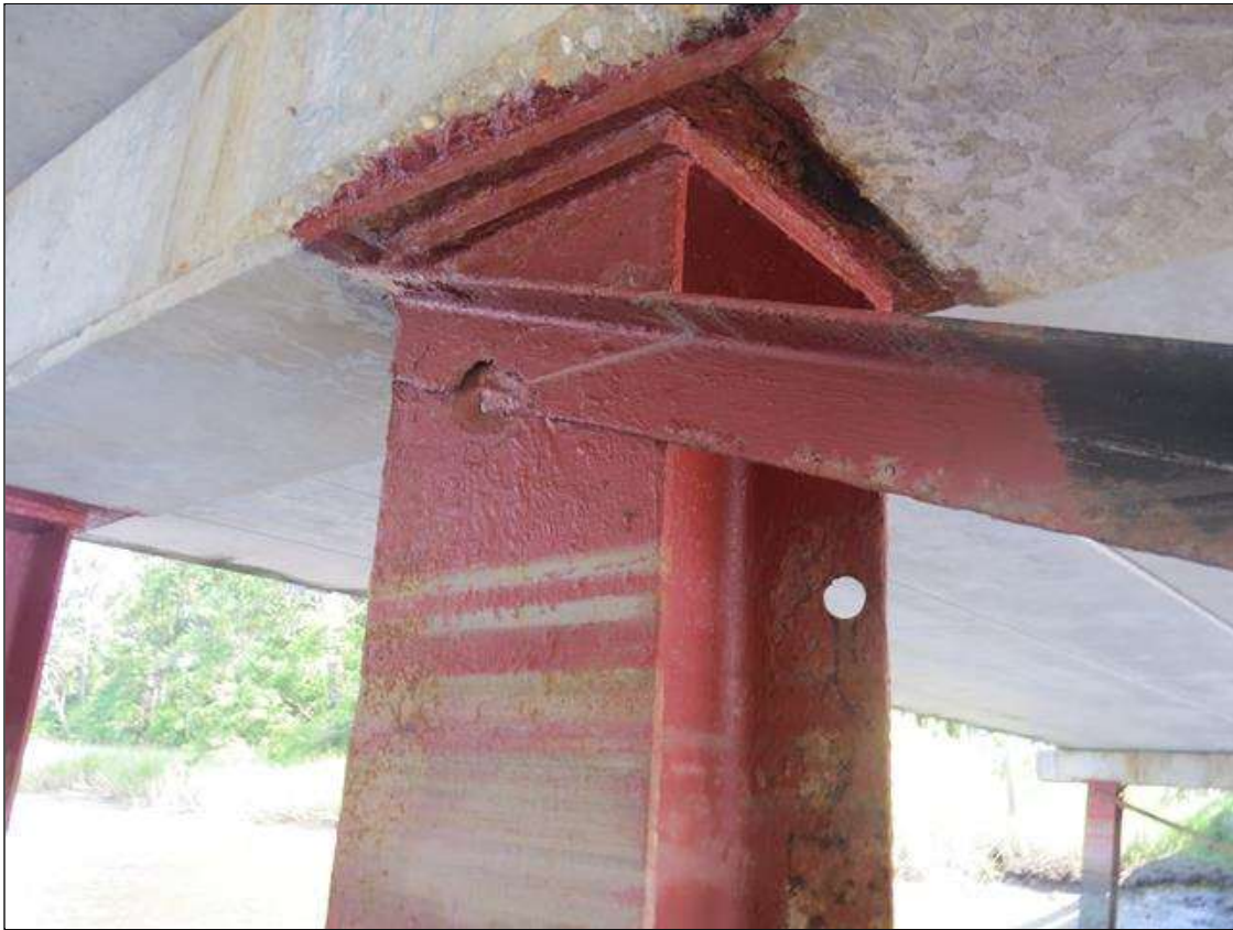
BENT 5 COLUMN 3 - 50% SECTION LOSS AT FAR RIGHT FLANGE AT 1.5IN DIAMETER HOLE LOCATION. 1/4IN TAPERED SECTION LOSS 1/4IN REMAINING AT NEAR LEFT. 1/8IN TAPERED SECTION LOSS 3/8IN REMAINING AT FAR LEFT FLANGE EDGE. (PAR PHOTO)
