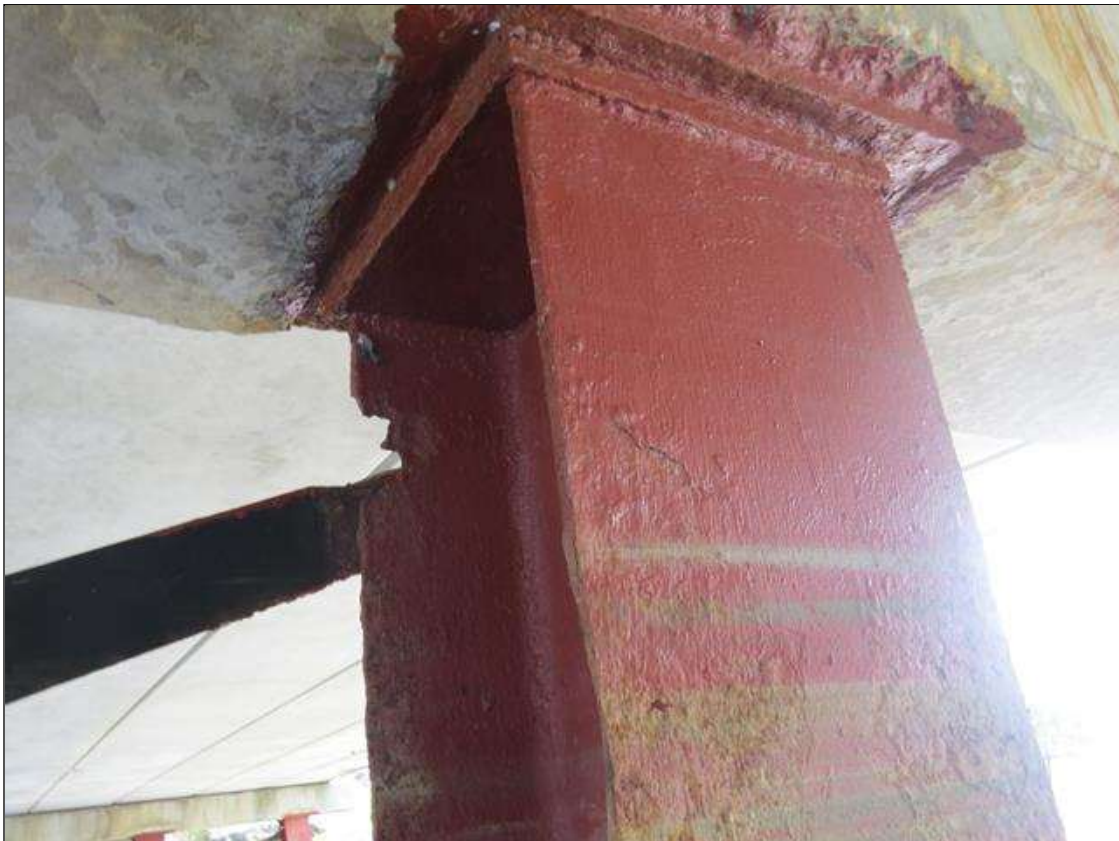
BENT 5 COLUMN 4 - 100% SECTION LOSS (2IN W X 3IN H) 6IN FROM TOP AT FAR LEFT FLANGE (PAR PHOTO)
