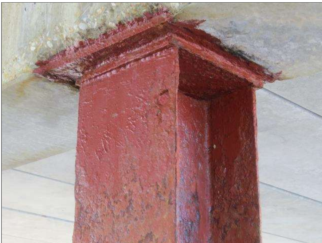
BENT 2 COLUMN 2 - 1/4IN TAPERED SECTION LOSS 1/4IN REMAINING TO LEFT FLANGES
