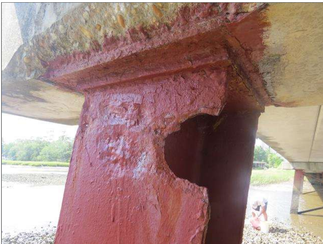
BENT 4 COLUMN 6 - 100% SECTION LOSS TO FAR LEFT FLANGE. KNIFE EDGED WITH UP TO 50% SECTION LOSS TO FAR RIGHT FLANGE. (PAR PHOTO)
