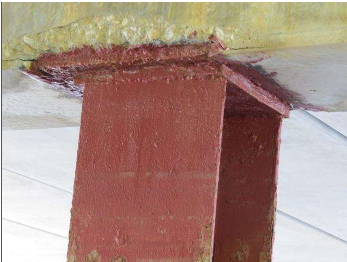
BENT 6 COLUMN 2 - 1/4IN TAPERED SECTION LOSS 1/4IN REMAINING AT ALL FLANGE EDGES TO FEET FROM TOP. (PAR PHOTO)
