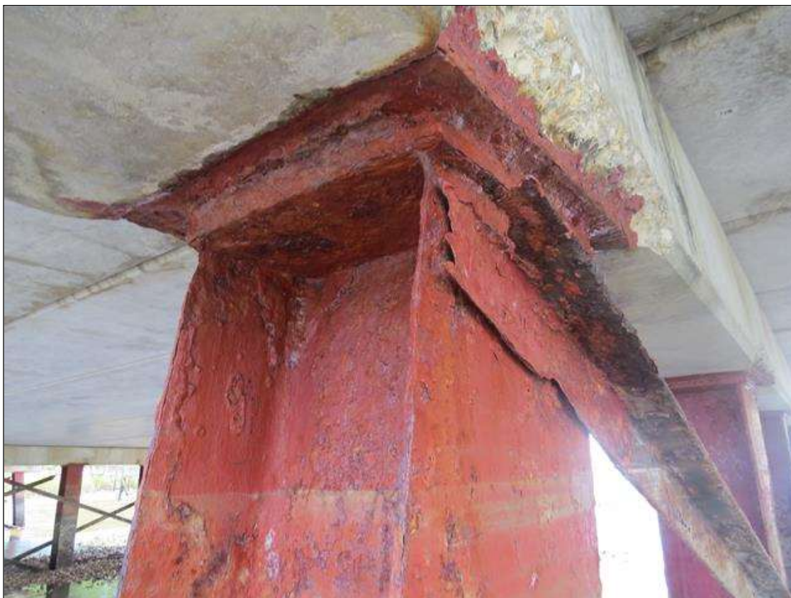
BENT 3 COLUMN 1 - 1/4IN FULL LENGTH SECTION LOSS, 1/4IN REMAINING AT TOP 2IN OF COLUMN AT LEFT FLANGE EDGES, 1/8IN SECTION LOSS ON LEFT SIDE. (PAR PHOTO)
