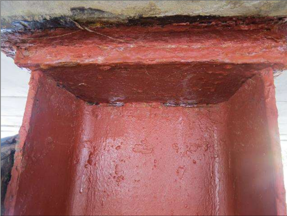
BENT 4 COLUMN 3 - 100% SECTION LOSS TO HALF OF THE WEB TO TOP CAP INTERFACE. 1/8IN TAPERED SECTION LOSS 3/8IN REMAINING AT ALL FLANGE EDGES. (PAR PHOTO)
