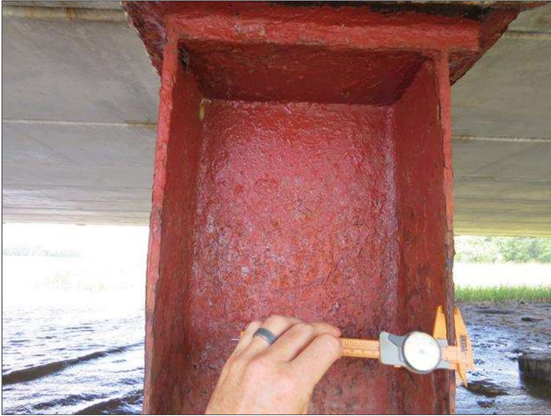
BENT 1 COLUMN 2 - UP TO 1/4IN TAPERED SECTION LOSS 1/4IN REMAINING AT ALL FLANGE EDGES. (PAR PHOTO)
