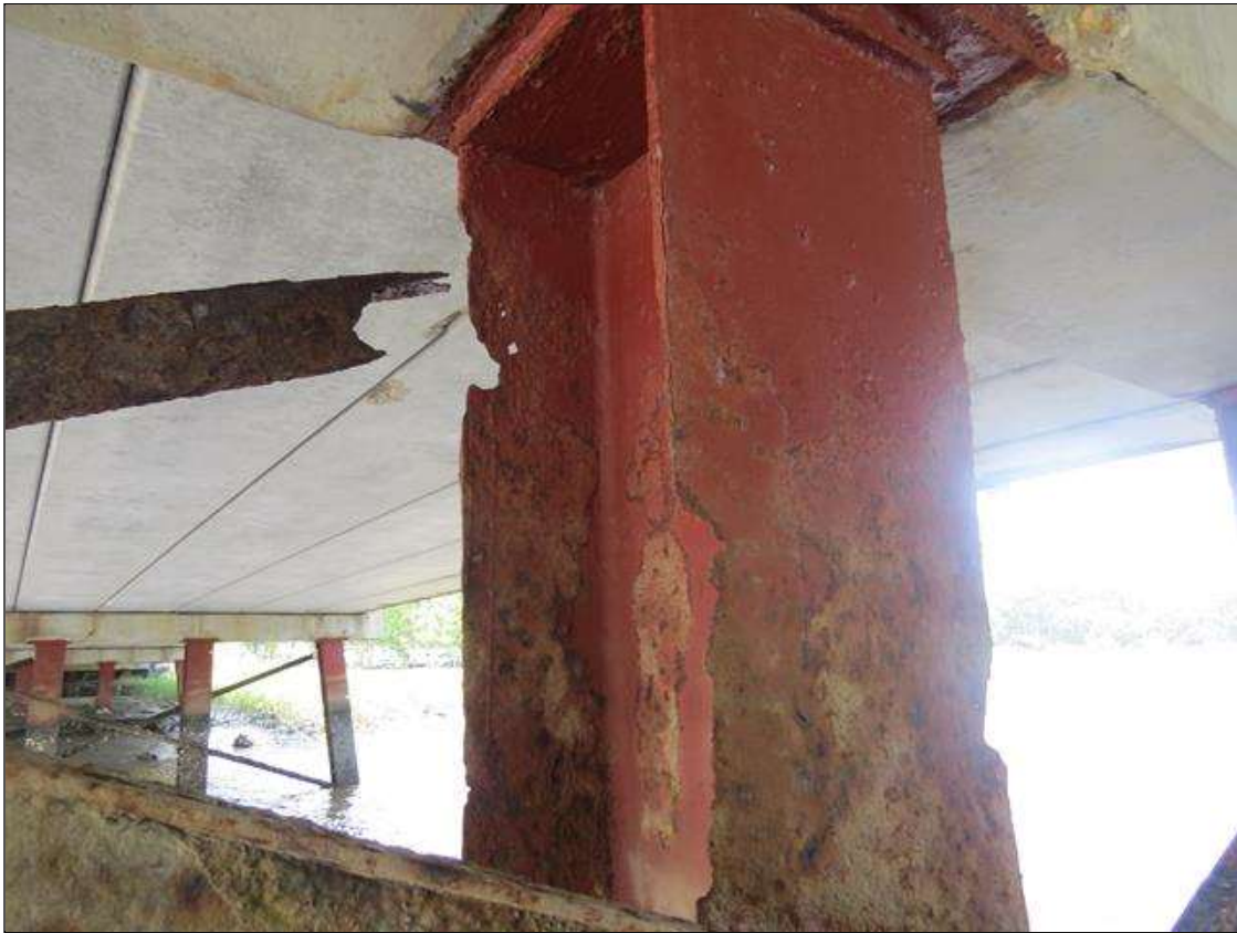
BENT 3 COLUMN 3 - 60% SECTION LOSS TO BOTH SIDES (UP TO 100% SECTION LOSS TO FLANGE EDGES FOR 2IN W X 12IN H) OF FAR FLANGE AND NEAR RIGHT FLANGE IN TOP 2FT OF COLUMN. 1/4IN TAPERED SECTION LOSS, 1/4IN REMAINING AT NEAR LEFT FLANGE EDGE 2FT FROM TOP. (PAR PHOTO)
