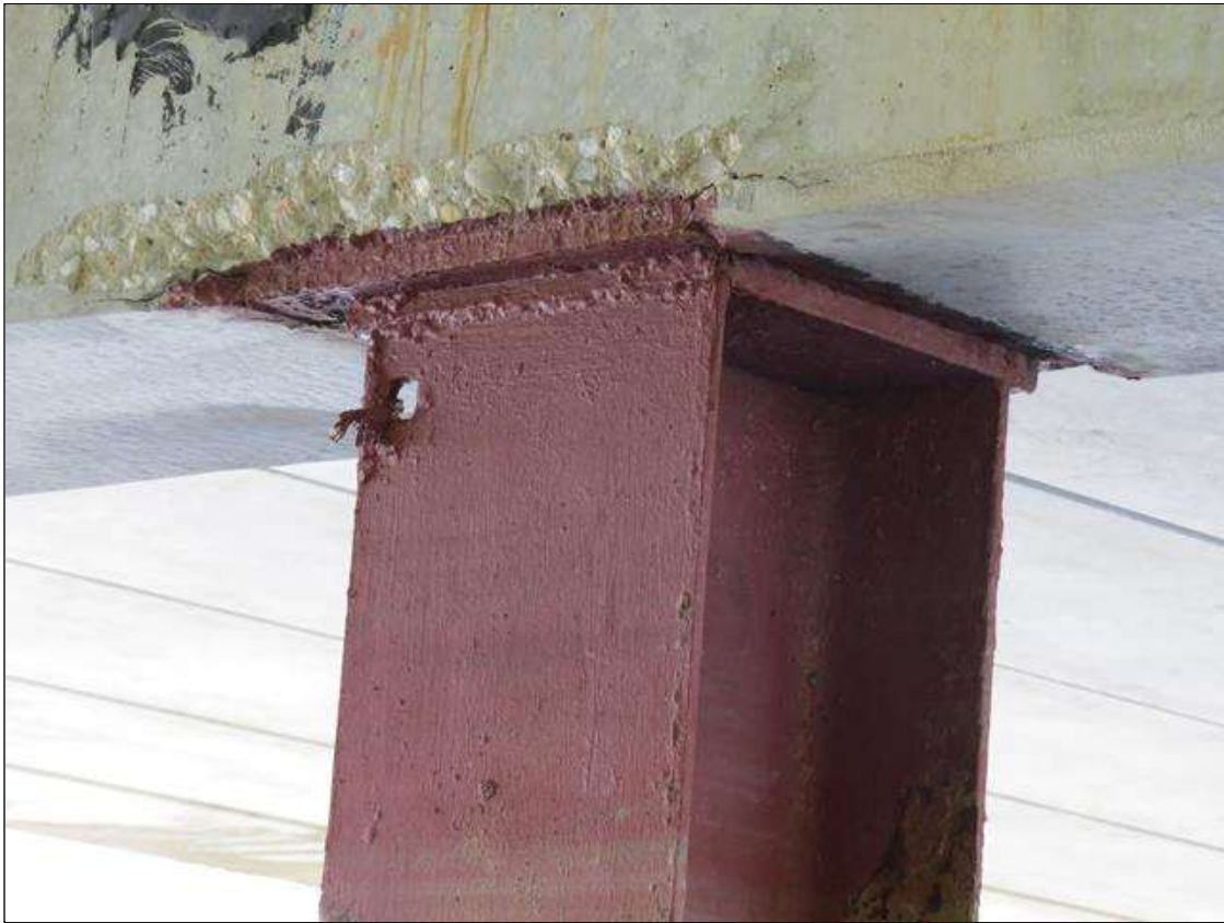
BENT 6 COLUMN 3 - 1/4IN TAPERED SECTION LOSS 1/4IN REMAINING AT ALL FLANGE EDGES 2FT FROM TOP. 1IN DIAMETER HOLE IN FAR RIGHT FLANGE. (PAR PHOTO)
