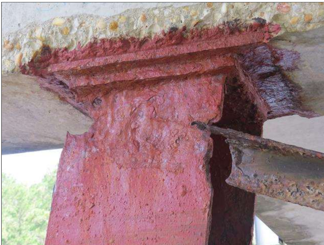
BENT 2 COLUMN 1 - UP TO 65% SECTION LOSS TO NEAR FLANGE, FAR FLANGE UP TO 50% SECTION LOSS ON LEFT SIDE. (PAR PHOTO)
