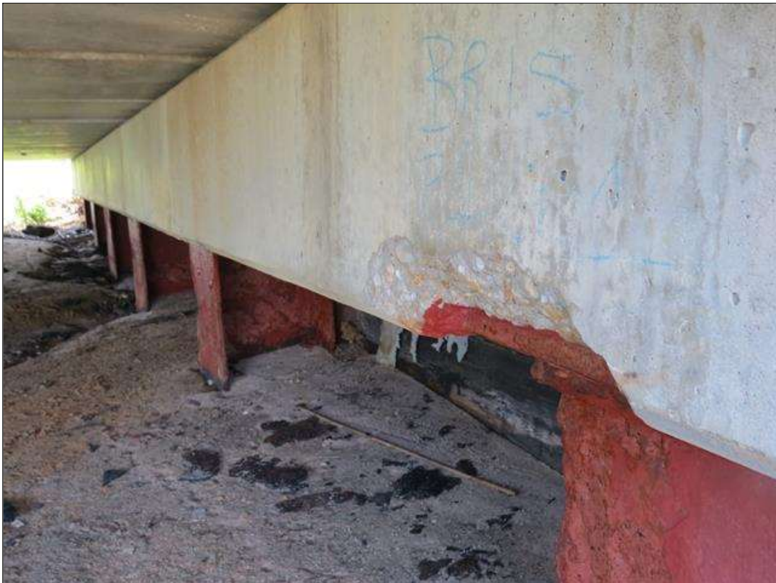
END BENT 1 CAP - SPALLS (14IN X 3IN X 1IN) TO BOTTOM OF CAP AT COLUMNS 1 & 6.
