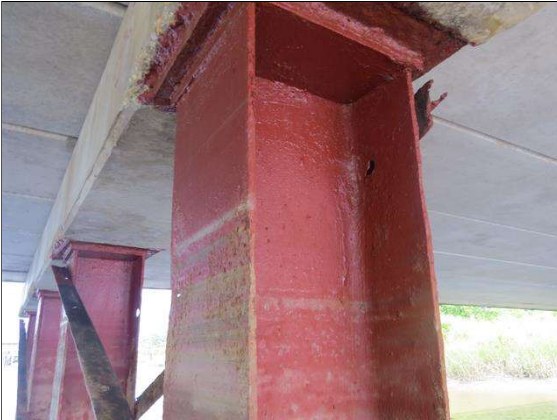
BENT 5 COLUMN 4 - KNIFE EDGING AT NEAR LEFT FLANGE WITH UP TO 50% SECTION LOSS. 1/4IN TAPERED SECTION LOSS 1/4IN REMAINING AT NEAR RIGHT FLANGE EDGE. (PAR PHOTO)
