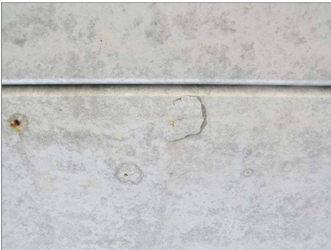
SPAN 2 BEAM 6 - MINOR DELAMINATION (5IN X 5IN) AT RIGHT SIDE AT MID-SPAN
