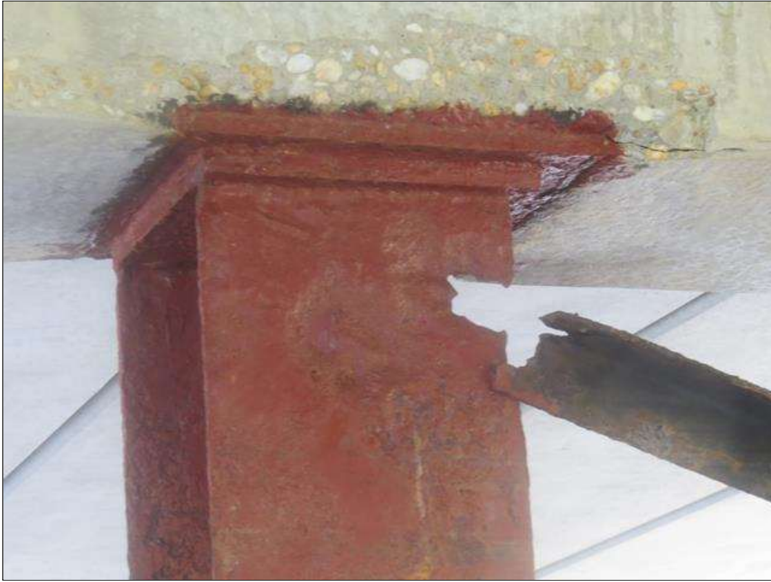
BENT 2 COLUMN 3 - 90% SECTION LOSS TO NEAR RIGHT FLANGE. 1/4IN TAPERED SECTION LOSS 1/4IN REMAINING TO NEAR LEFT FLANGE. 1/8IN TAPERED SECTION LOSS 3/8IN REMAINING AT FAR FLANGES. (PAR PHOTO)
