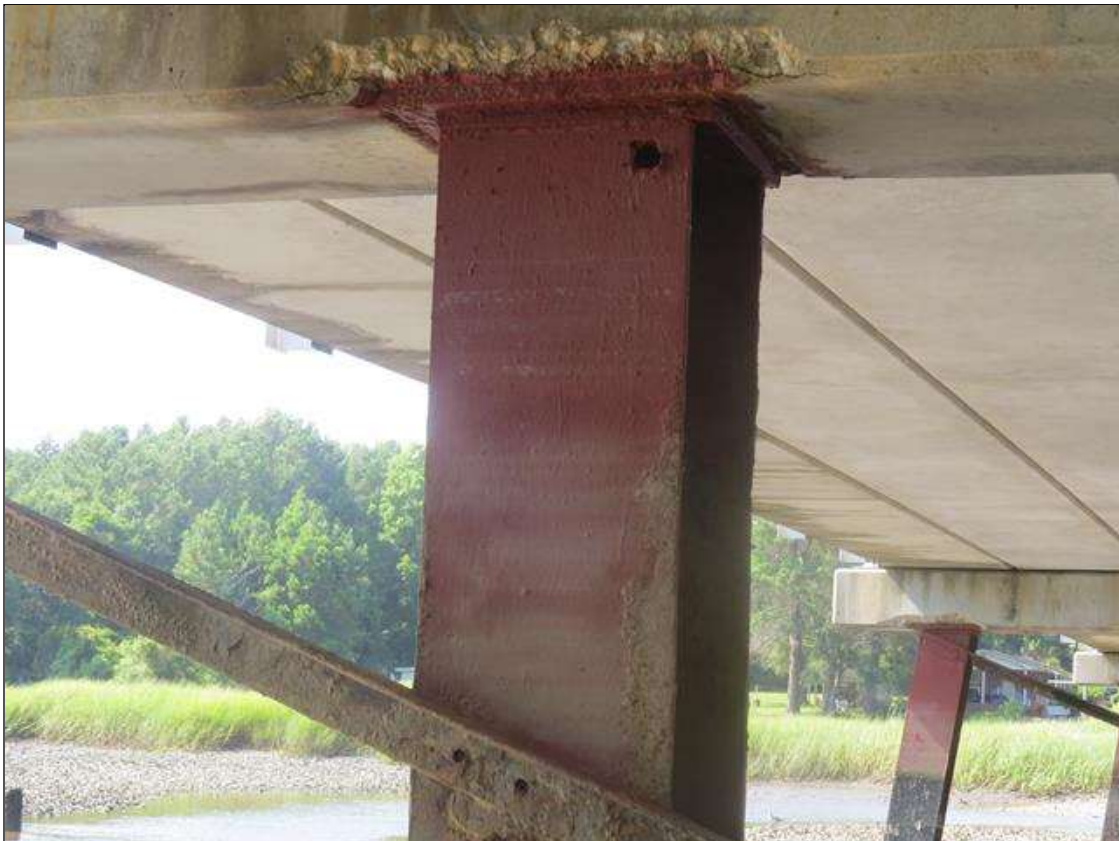
BENT 6 COLUMN 5 - 1/8IN TAPERED SECTION LOSS 3/8IN REMAINING AT ALL FLANGE EDGES. 1IN DIAMETER HOLE AT FAR LEFT AT TOP.
