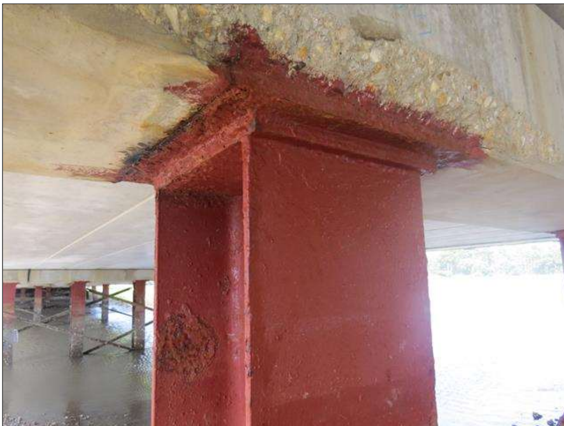
BENT 4 COLUMN 5 - KNIFE EDGING TO FAR RIGHT FLANGE. 1/4IN TAPERED SECTION LOSS 1/4IN REMAINING AT BOTH LEFT FLANGE EDGES. (PAR PHOTO)
