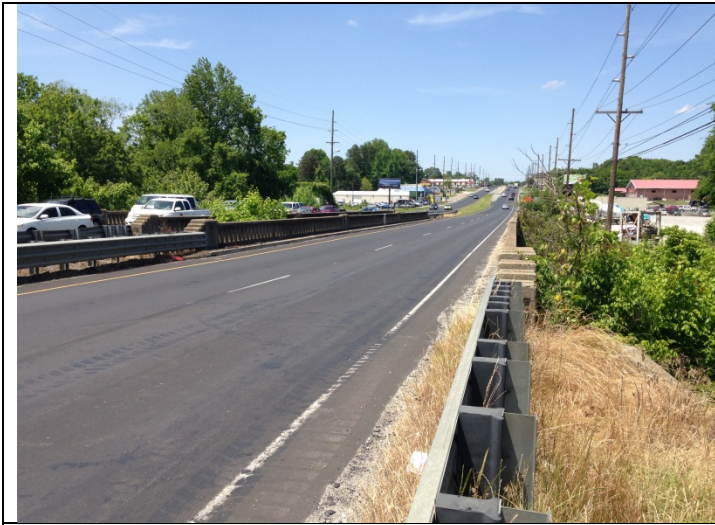
Bridge 57 on US 29 & US 601 over Irish Buffalo Creek. View to the north.
