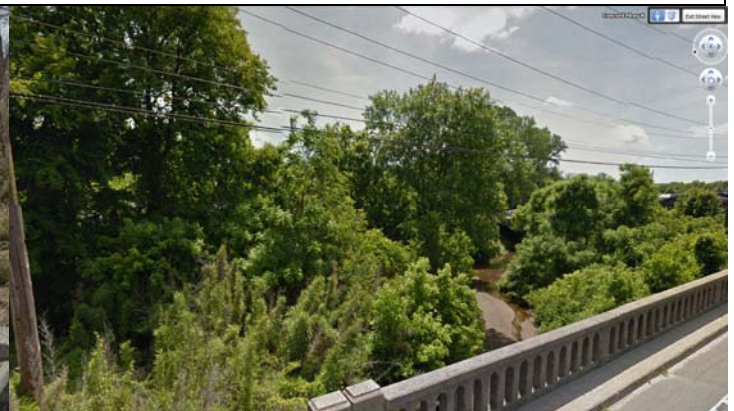
Bridge 59 on US 29 & US 601 view of Irish Buffalo Creek southeastward. (Google Streetview c. 2015)
