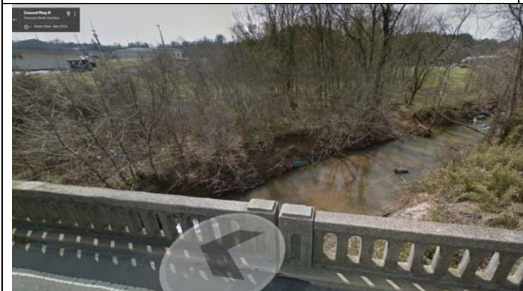
Bridge 57 on US 29 & US 601 view of Irish Buffalo Creek northwestward. (Google Streetview c. 2015)
