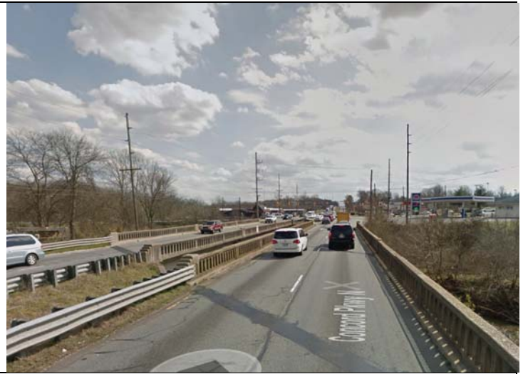
Bridges 57 (left) & 59 (right) on US 29 & US 601 over Irish Buffalo Creek. View to the south. (Google Streetview c. 2015)
