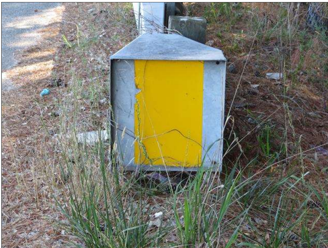
TERMINAL GUARDRAIL END
