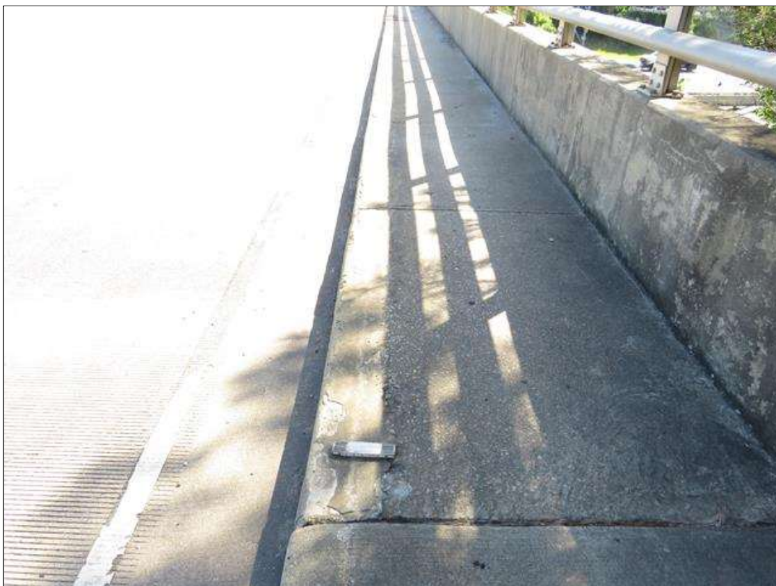
Span 1 Right Bridge Rail: SCATTERED SCALING UP TO 1/8" DEEP ALONG FACE OF CURB AT NEAR END.
