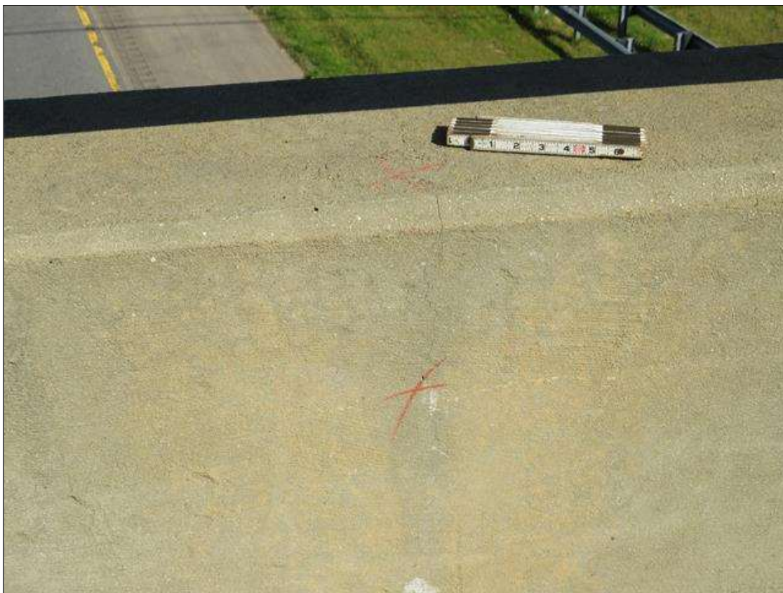
Span 1 Left Bridge Rail: PARTIAL DEPTH VERTICAL HAIRLINE TO OPEN (1/32") CRACKING IN BRIDGE RAILING. FULL HEIGHT VERTICAL HAIRLINE CRACKS WITH LIGHT EFFLORESCENCE IN NEGATIVE MOMENT REGION, 4 TOTAL
