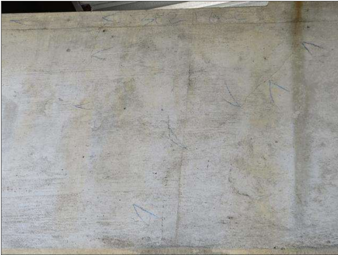
Bent 1 Cap 1: CRACKING ON BOTH FACES OVER COLUMN 1 & 6, HAIRLINE to 1/64" WIDE CRACKS ARE DIAGONAL AND VERTICAL, RUNNING FROM TOP EDGE DOWN TOWARDS BOTTOM EDGE. MINOR HAIRLINE CRACK AT BOTTOM OF CAP BETWEEN COLUMNS 5 & 6
