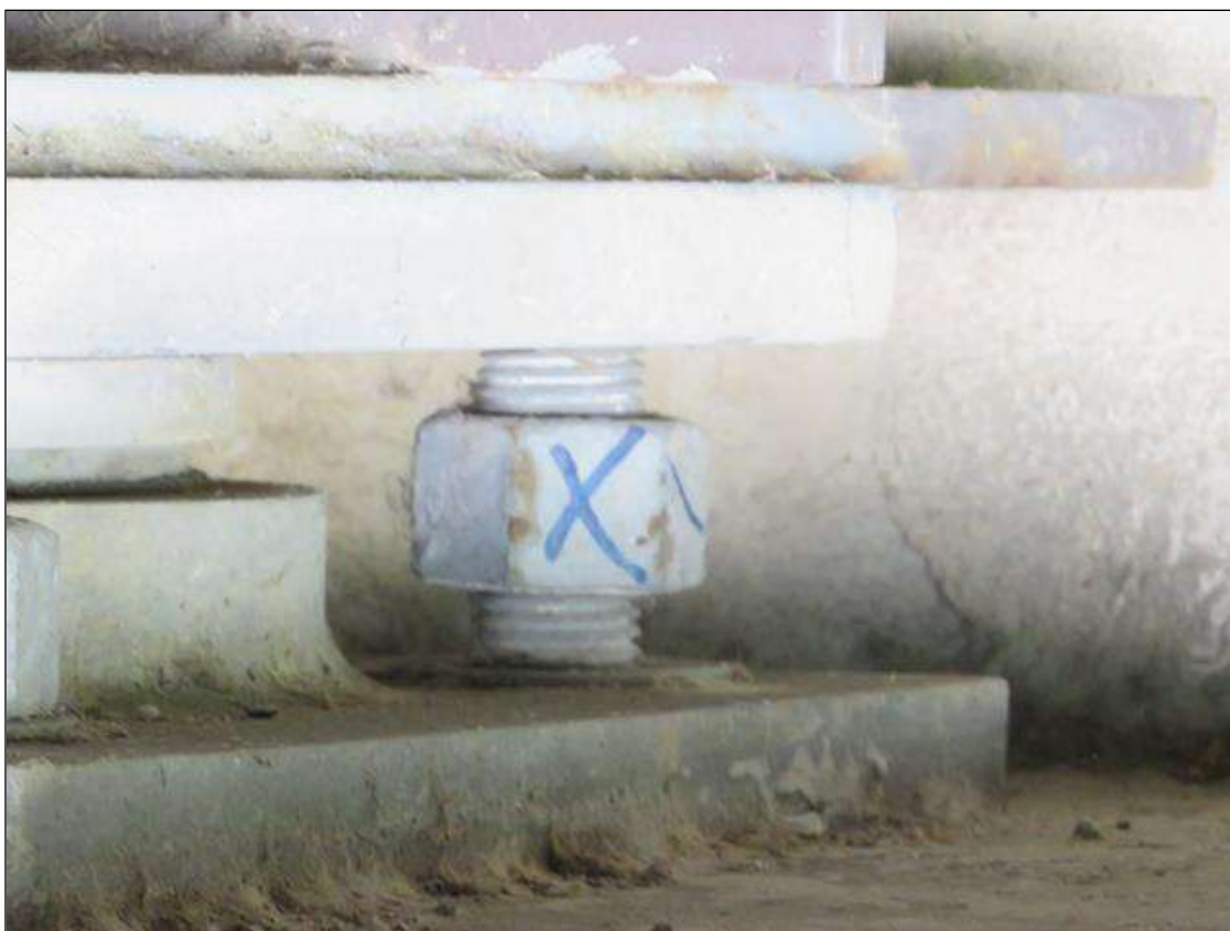
Span 1 Beam 9 - Far Bearing: SPAN 1 BEAM 9 FAR BEARING (1) OF (4) CONNECTION NUTS LOOSE [REAR]
