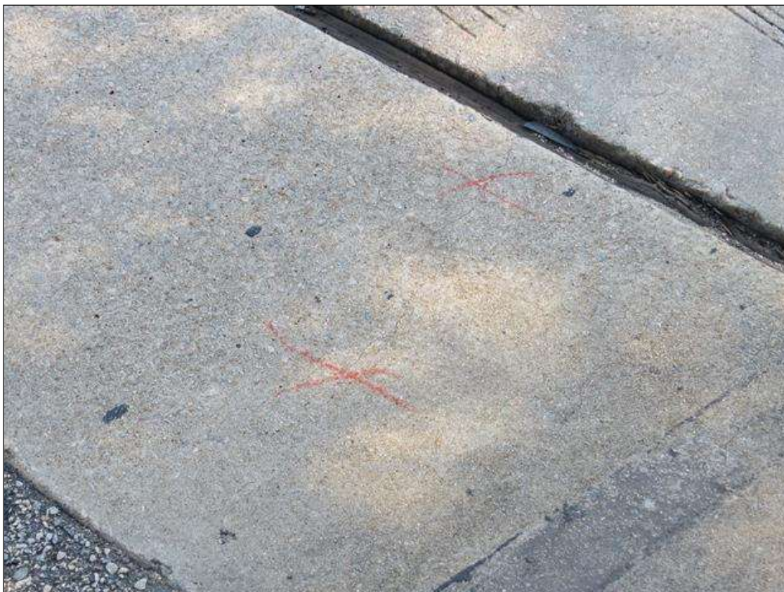
Approach 1 : SCATTERED ACROSS THE WIDTH, FULL LENGTH LONGITUDINAL CRACKING TO 1/32" WIDE
