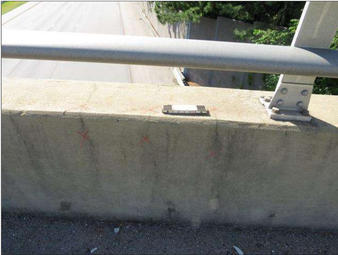
Span 1 Right Bridge Rail: FULL HEIGHT VERTICAL HAIRLINE CRACKING IN RIGHT BRIDGE RAILING IN NEGATIVE MOMENT REGION
