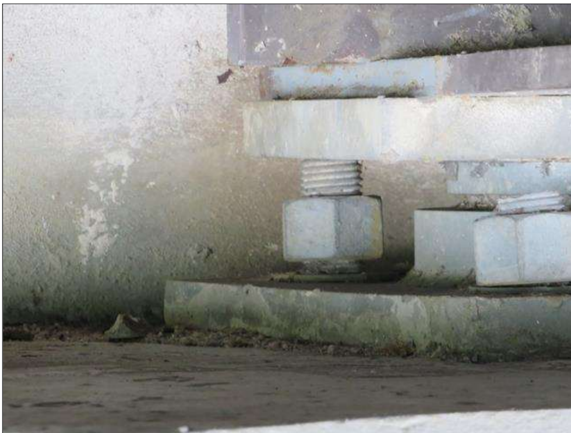
Span 1 Beam 3 - Far Bearing: SPAN 1 BEAM 3 FAR BEARING(1) OF (4) CONNECTION NUTS LOOSE [REAR]
