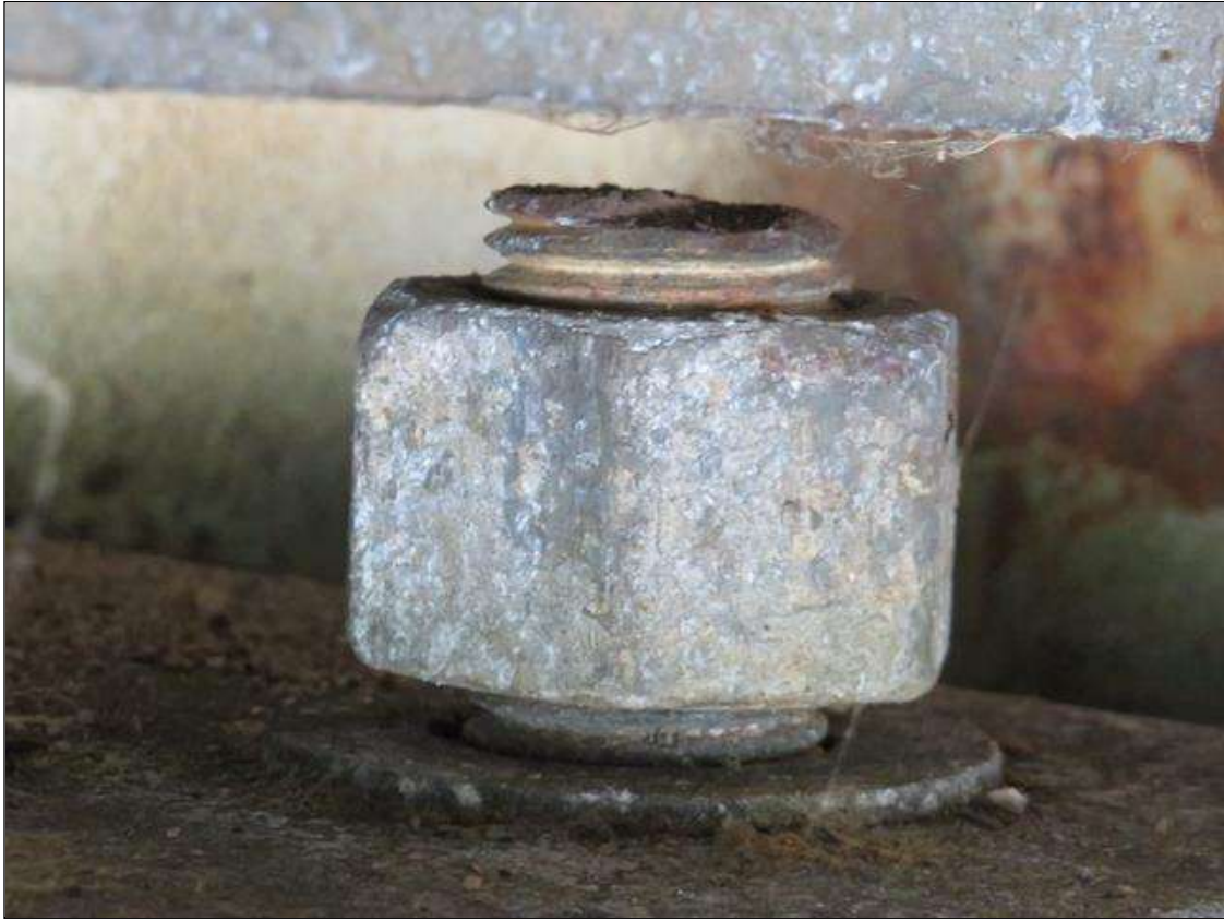
Span 1 Beam 10 - Near Bearing: SPAN 1 BEAM 10 (1) OF (4) ANCHOR NUTS LOOSE [REAR]
