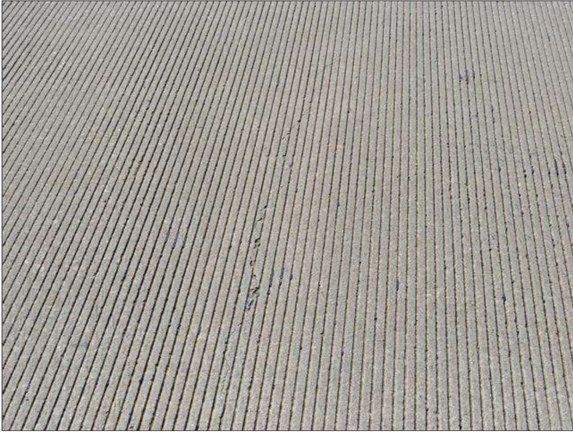
Span 2 Deck: TOP OF THE DECK AT THE SOUTH END, SCATTERED ACROSS THE WIDTH, LONGITUDINAL CRACKING TO 1/64" WIDE EMANATES FROM THE JOINT HEADER, AND TRANSVERSE CRACKING TO 1/64" WIDE SCATTERED THROUGHOUT; UNDERSIDE OF THE OVERHANGS, SCATTERED HAIRLINE TRANSVERSE CRACKING WITH SOME EFFLORESCENCE
