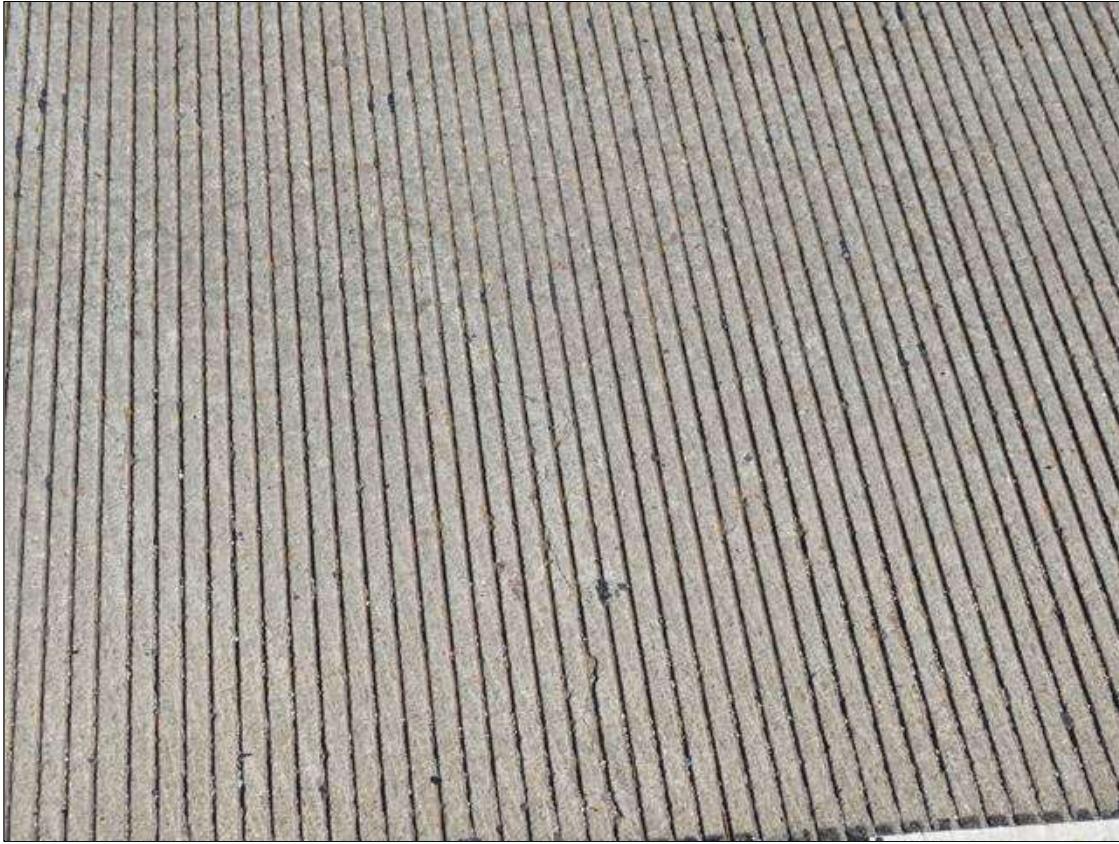
Span 1 Deck: TOP OF THE DECK AT THE SOUTH END, SCATTERED ACROSS THE WIDTH, LONGITUDINAL CRACKING TO 1/64" WIDE EMANATES FROM THE JOINT HEADER, AND TRANSVERSE CRACKING TO 1/64" WIDE SCATTERED THROUGHOUT; UNDERSIDE OF THE OVERHANGS, SCATTERED HAIRLINE TRANSVERSE CRACKING WITH SOME EFFLORESCENCE
