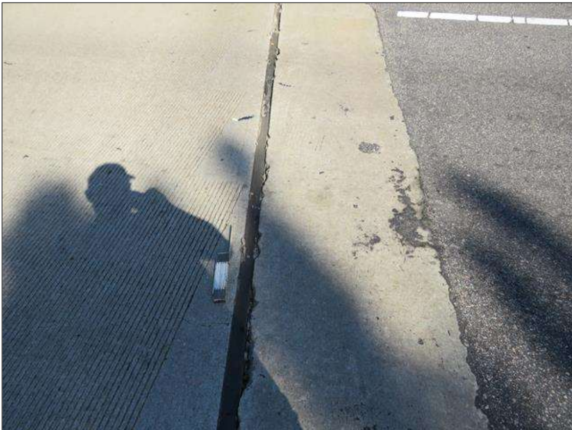
Span 2 Expansion Joint: ADJACENT DECK HEADERS, SCATTERED ALONG THE LENGTH, EDGE CHIPPING [UP TO 1" WIDE X 1" DEEP] ALONG END BENT 2 JOINT.
