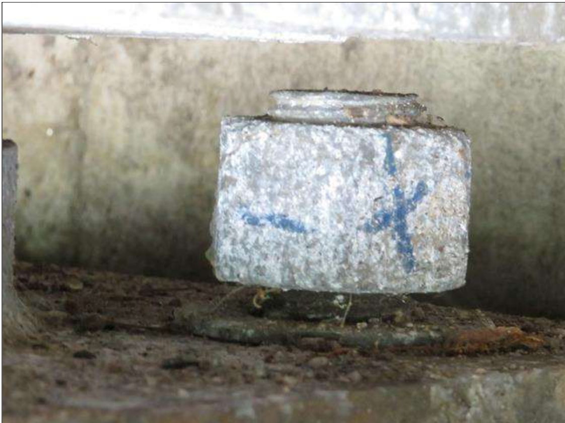
Span 1 Beam 5 - Near Bearing: (1) OF (4) SPAN 1 BEAM 5 NEAR ANCHOR NUTS LOOSE [REAR]
