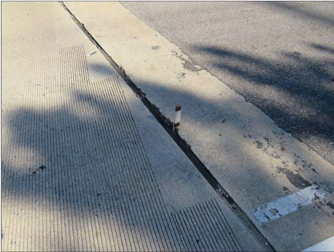
Span 2 Expansion Joint: SEAL ADHESION FAILURE, SCATTERED LEAKING THROUGHOUT END BENT 2 JOINT.
