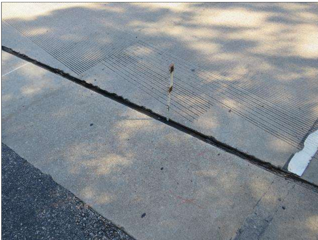
Span 1 Expansion Joint: 50% ADHESION LOSS OF DECK JOINT. JOINT LEAKING AT BAYS 8, 9, 12, 13 AT END BENT 1.
