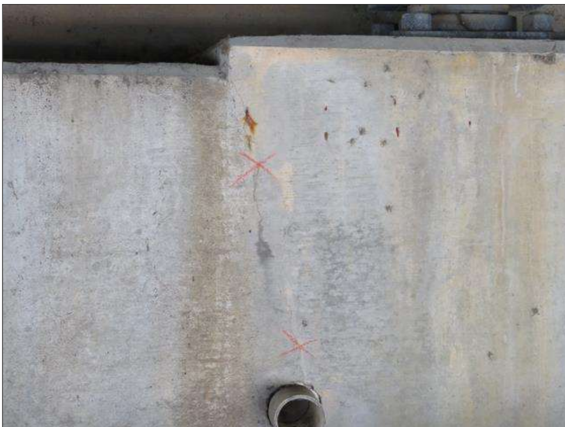
End Bent 2 CAP: (10) SCATTERED VERTICAL HAIRLINE CRACKS UP TO 1' HIGH.
