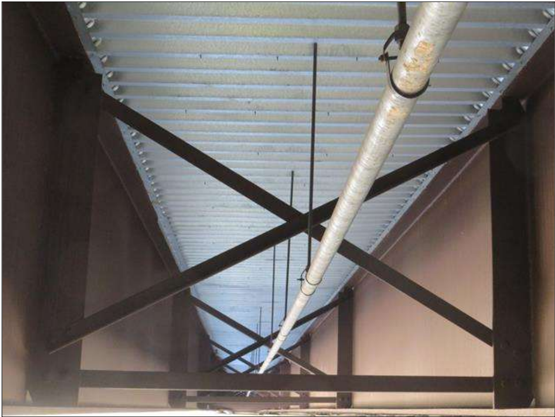
UTILITY BAY 1 1.5" STEEL PIPE
