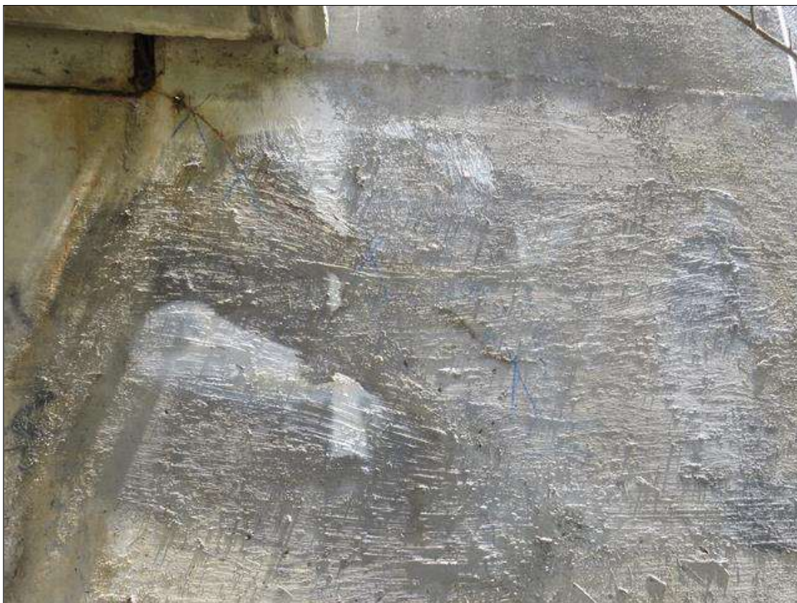
End Bent 2 Abutment: 2 DIAGONAL HAIRLINE CRACKS (2' EACH) AT LEFT AND RIGHT SIDE ABUTMENT EXTENSIONS, FULL HEIGHT VERTICAL AND DIAGONAL HAIRLINE CRACKS
