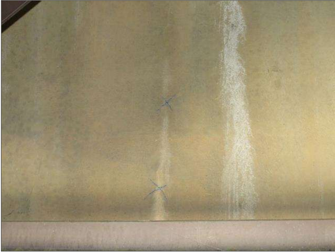
End Bent 1 Abutment: VERTICAL HAIRLINE TO 1/64" WIDE CRACK, FULL HEIGHT IN BAY 3, 9, 10 11 & 12. LONGITUDINAL HAIRLINE CRACK TO 1/64" WIDE IN TOP OF BACKWALL (12 TOTAL)
