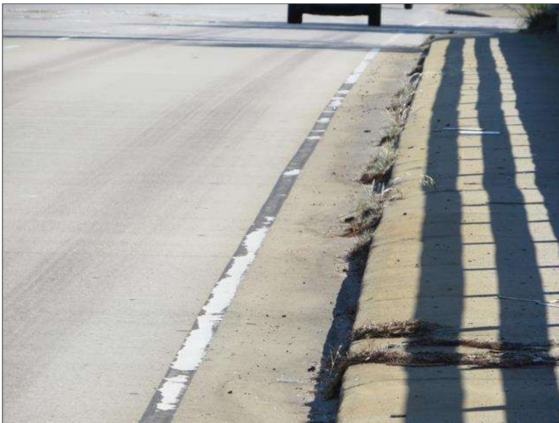
DECK DEBRIS UP TO 4" WIDE X 1" DEEP ALONG BOTH SHOULDERS
