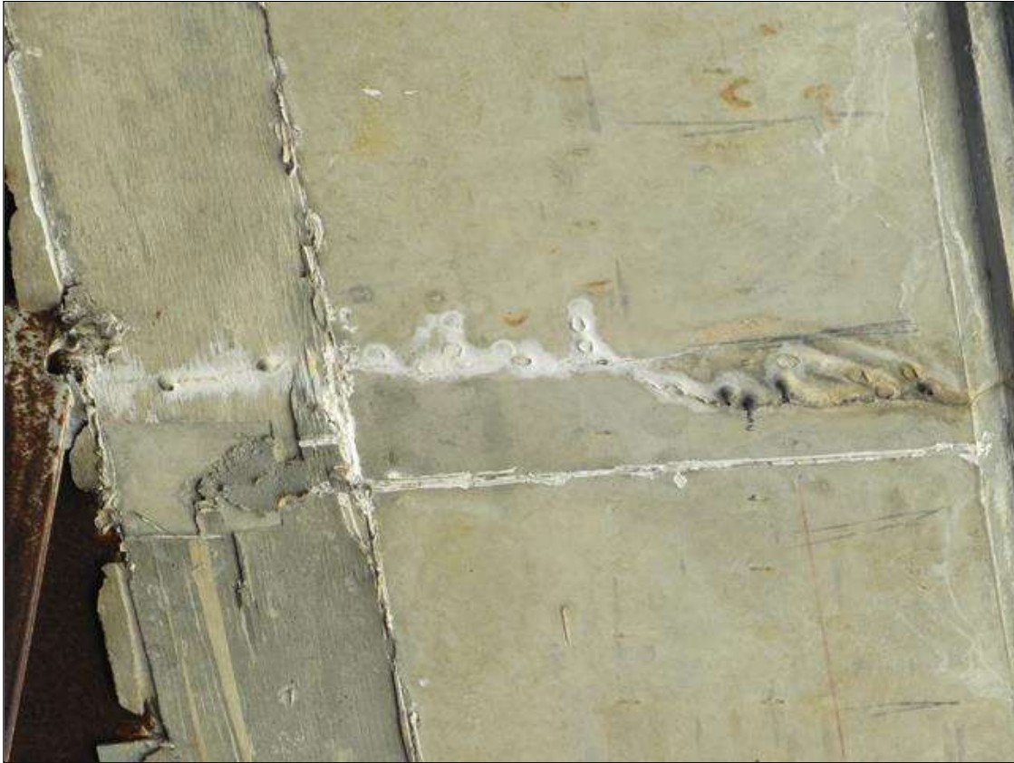
Span 1 Deck: TOP OF THE DECK AT THE SOUTH END, SCATTERED ACROSS THE WIDTH, LONGITUDINAL CRACKING TO 1/64" WIDE EMANATES FROM THE JOINT HEADER, AND TRANSVERSE CRACKING TO 1/64" WIDE SCATTERED THROUGHOUT; UNDERSIDE OF THE OVERHANGS, SCATTERED HAIRLINE TRANSVERSE CRACKING WITH SOME EFFLORESCENCE
