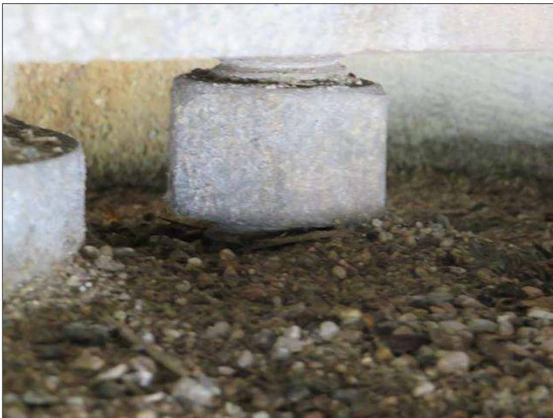
Span 1 Far Bearing: SPAN 1 BEAM 5 FAR BEARING(1) OF (4) ANCHOR NUTS LOOSE [REAR]
