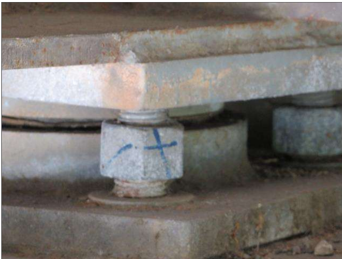
Span 1 Beam 13 - Far Bearing: SPAN 1 BEAM 13 FAR BEARING (1) OF (4) CONNECTION NUTS LOOSE [NEAR]
