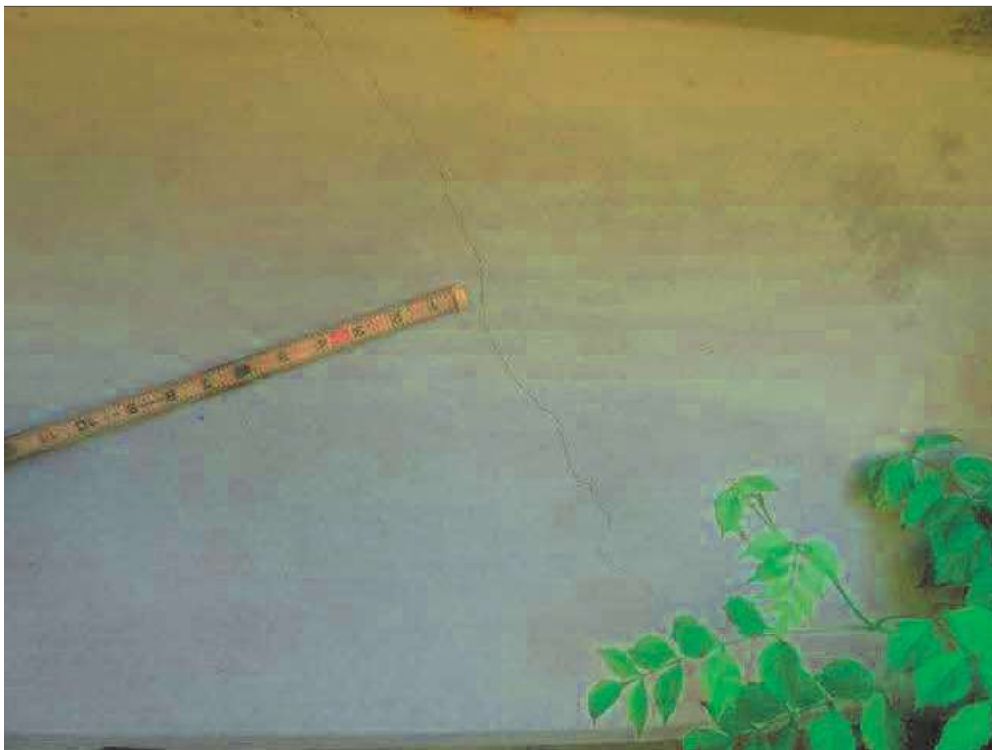
Span 1 Beam 1: 6' SECTION OF UP TO 0.012" DIAGONAL CRACKS IN LEFT FACE OF GIRDER EXTENDING FROM ABUTMENT 1, CRACK APPROXIMATELY 18" FROM ABUTMENT 1 SHOWN
