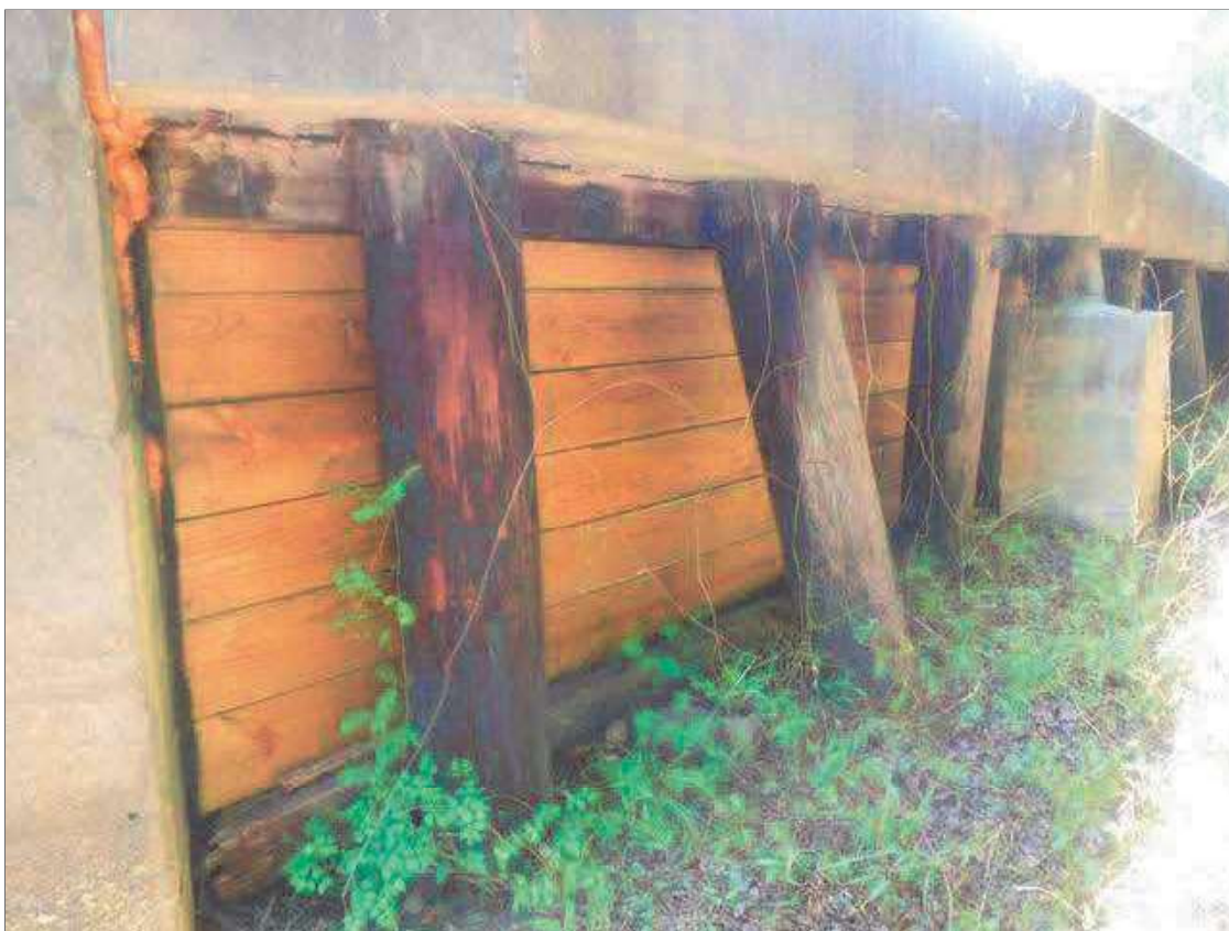
PRIORITY MAINTENANCE REPAIR TO SOUTHEAST WINGWALL SINCE 2018 INSPECTOIN
