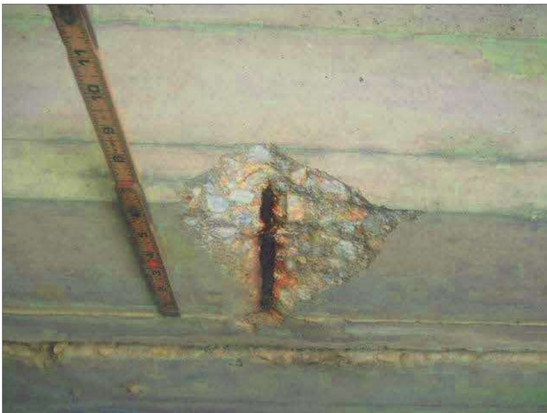
Span 4 Beam 1: 8" X 5" X 1" DEEP SPALL WITH EXPOSED REBAR IN BOTTOM OF PIER 3 DIAPHRAGM IN BAY 1
