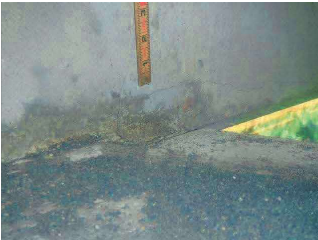
Span 2 Beam 2: 16" X 4" X 4" AREA OF DELAMINATION WITH UP TO 0.025" LONGITUDINAL AND HORIZONTAL CRACKS IN BOTTOM AND RIGHT FACE OF GIRDER AT PIER 1
