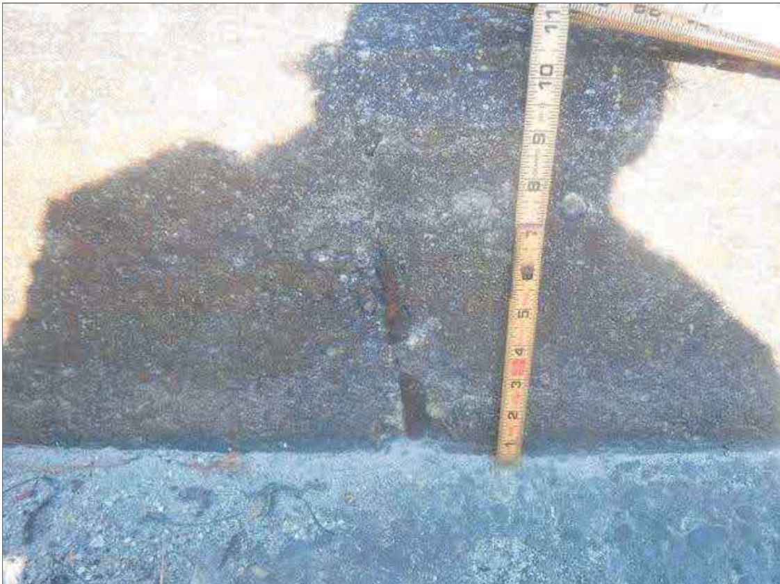
Span 2 Right Bridge Rail: (3) AREAS OF EXPOSED REBAR UP TO 7" X 1" IN FACE OF RAIL APPROXIMATELY 7', 12', AND 13' FROM PIER 1 JOINT, CONDITION 12' FROM PIER 1 JOINT SHOWN
