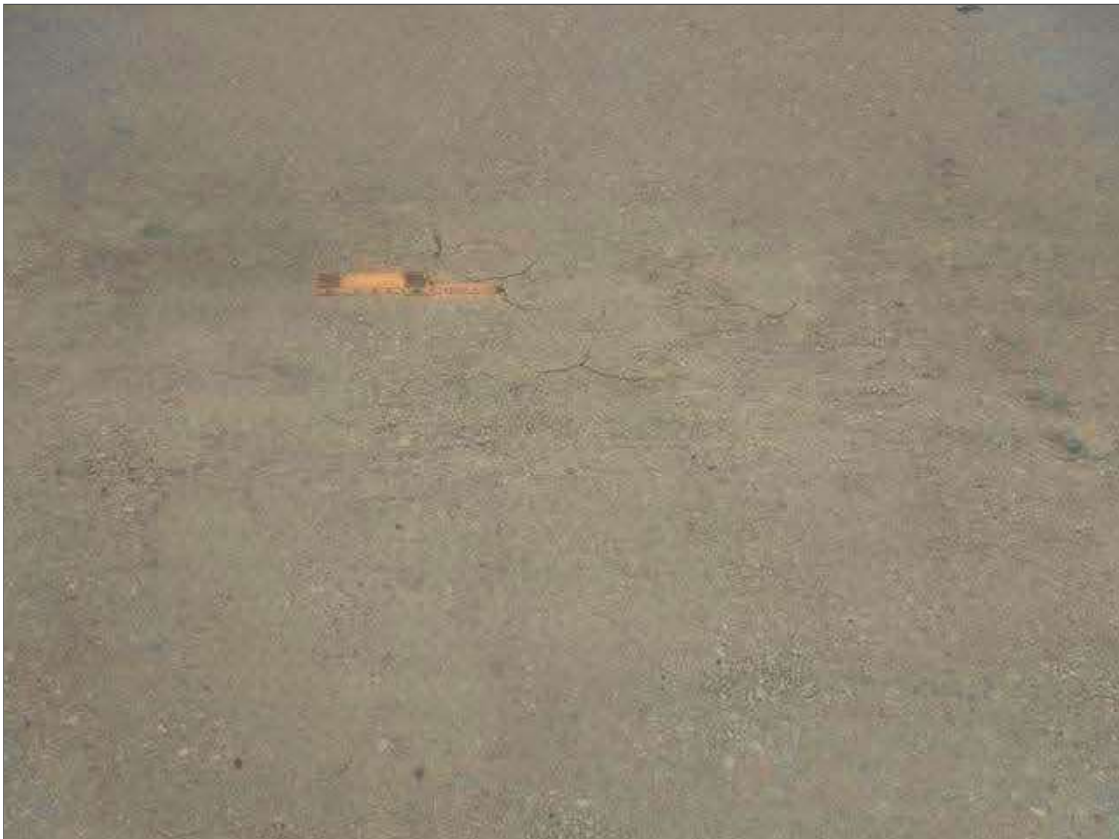
Span 3 Deck: UP TO 1/16" MAP CRACKS IN TOP OF DECK PRIMARILY IN TRAVEL LANES
