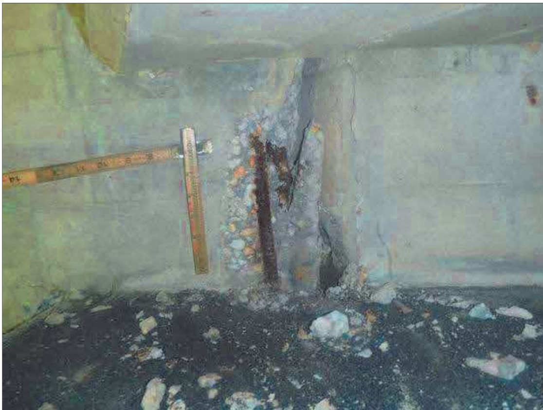
Span 1 Beam 3: PAR: 11" X 6" X 3" DEEP SPALL WITH EXPOSED REBAR IN RIGHT FACE OF GIRDER AT PIER 1
