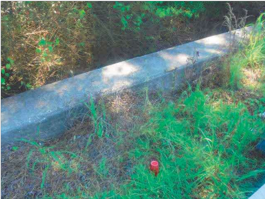
(2) AREAS OF SHOULDER EROSION UP TO 55" X 26" X 21" DEEP BEHIND SOUTHEAST WINGWALL, APPROXIMATELY 20' AND 24' FROM ABUTMENT 2 FILL FACE
