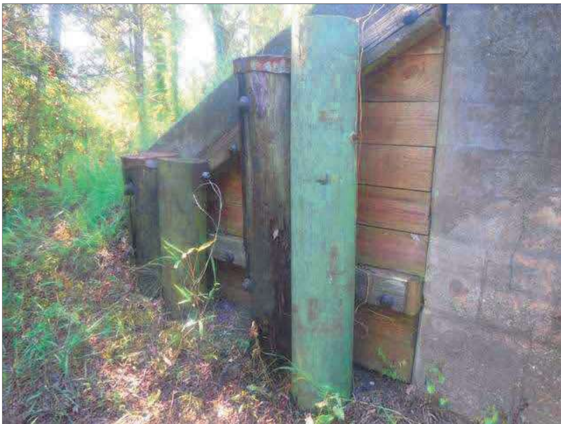
PRIORITY MAINTENANCE REPAIR TO SOUTHWEST WINGWALL SINCE 2018 INSPECTOIN
