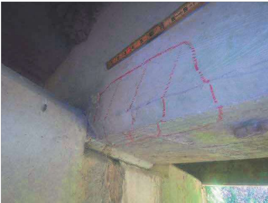
Span 1 Beam 3: 12" X 4" X 5" AREA OF DELAMINATION WITH UP TO 0.02" LONGITUDINAL AND HORIZONTAL CRACKS IN BOTTOM AND LEFT FACE OF GIRDER AT PIER 1
