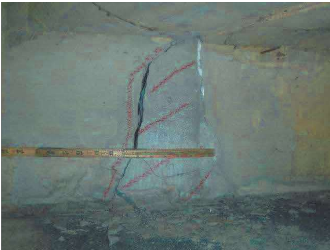
Span 3 Beam 2: 13" X 8" FAILED REPAIR WITH UP TO 1/4" DIAGONAL CRACK IN RIGHT FACE OF GIRDER AT PIER 3
