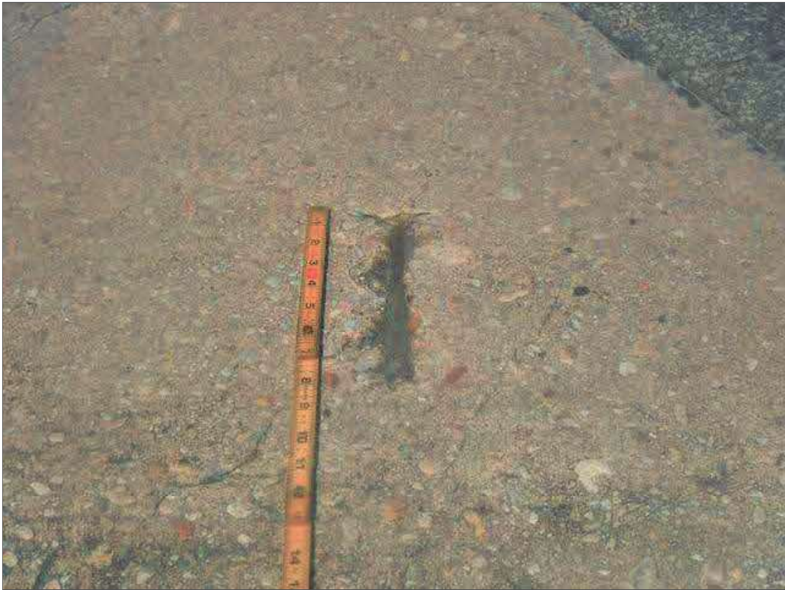
Span 4 Deck: PAR: 8" X 3" X 1/2" DEEP SPALL WITH EXPOSED REBAR IN TOP OF DECK IN WHEEL LINE OF EASTBOUND LANE, APPROXIMATELY 16" FROM ABUTMENT 2 FILL FACE
