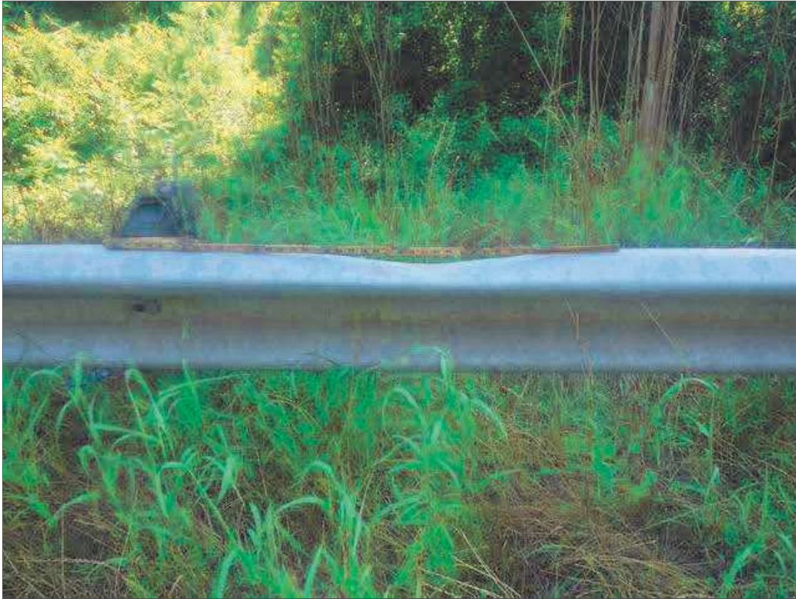
(2) AREAS OF DISTORTION UP TO 33" LONG X 2" ALONG TOP OF NORTHEAST APPROACH GUARDRAIL, APPROXIMATELY 23' AND 32' FROM ABUTMENT 2 FILL FACE, CONDITION APPROXIMATELY 32' FROM ABUTMENT 2 FILL FACE SHOWN; PREVIOUSLY NOTED IN SPAN 4 RIGHT RAIL
