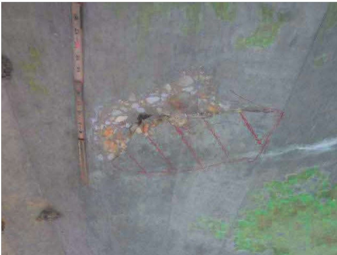
Span 1 Deck: 13" X 4" X 1" DEEP SPALL WITH EXPOSED REBAR AND 16" X 7" AREA OF DELAMINATION WITH UP TO 0.02" MAP CRACKS IN BOTTOM OF DECK IN BAY 1, APPROXIMATELY 7' FROM ABUTMENT 1
