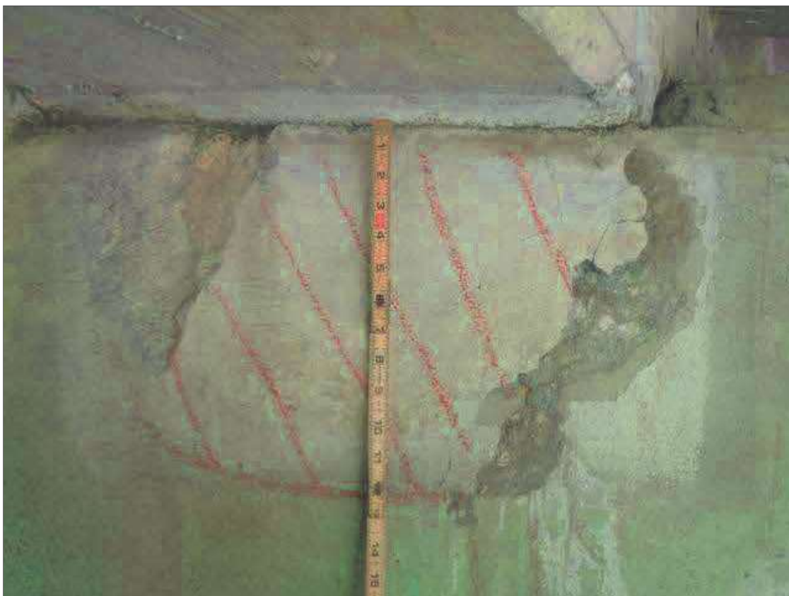
Bent 1 Cap 1: 21" X 12" FAILED REPAIR WITH UP TO 0.012" MAP CRACKS AND (2) SPALLS UP TO 12" X 4" X 1/2" DEEP IN SPAN 1 FACE OF CAP BENEATH GIRDER 3
