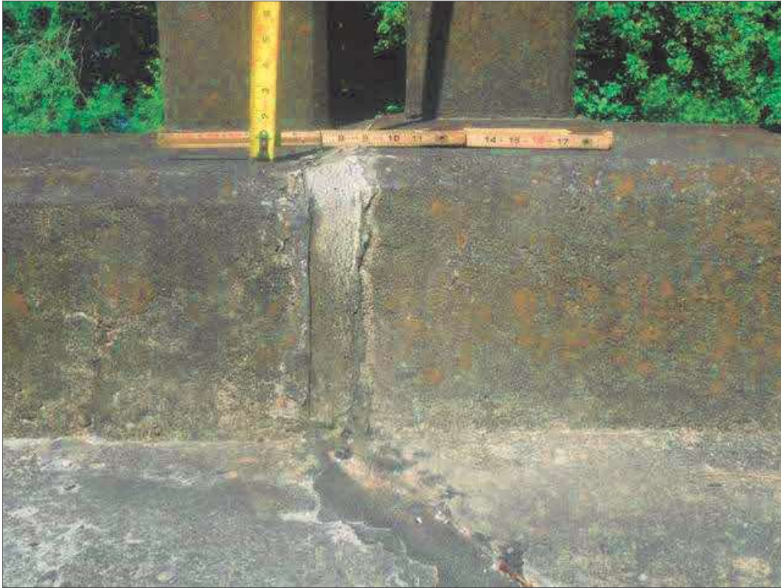
Span 2 Deck: UP TO 1/2" VERTICAL MISALIGNMENT BETWEEN SPAN 2 AND 3 DECKS ALONG PIER 2 JOINT, CONDITION AT LEFT CURB SHOWN
