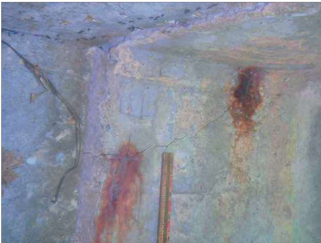
Span 2 Beam 4: UP TO 0.025" DIAGONAL CRACKS WITH RUST STAINING AND 2" X 1" AREA OF EXPOSED REBAR IN RIGHT FACE OF GIRDER AT PIER 1
