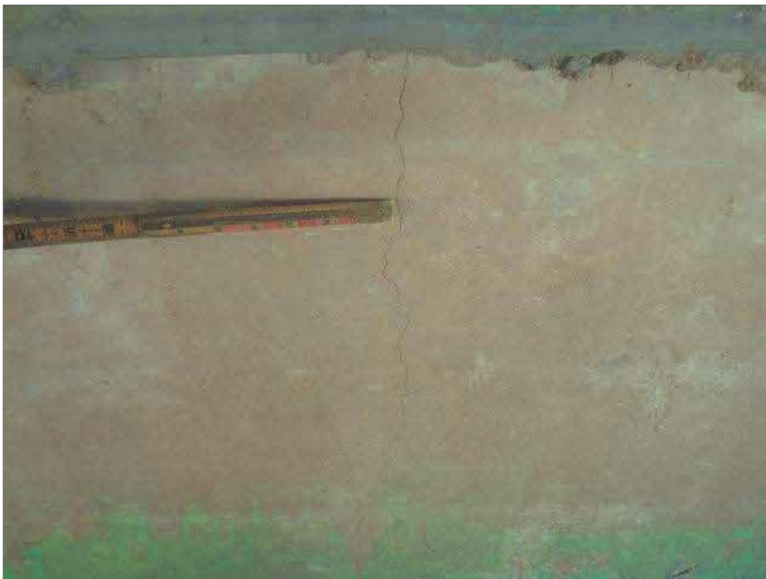
End Bent 1 Abutment: UP TO 0.016" VERTICAL CRACKS IN FACE OF ABUTMENT IN VARIOUS LOCATIONS, CRACK BENEATH BAY 2 SHOWN
