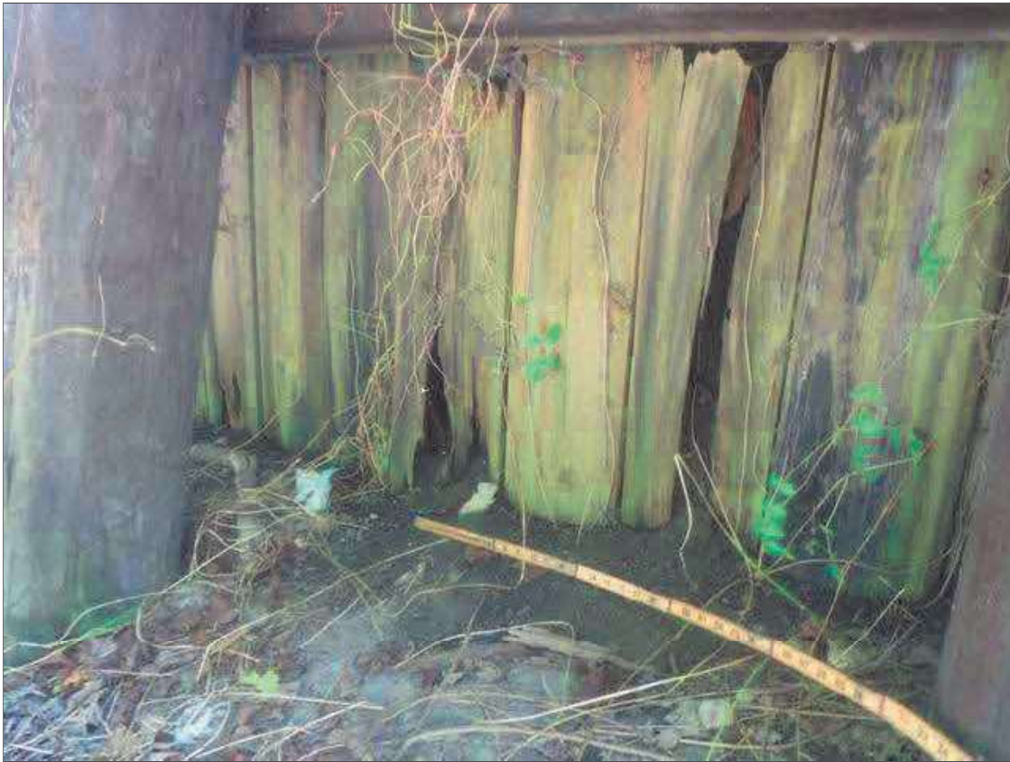
PAR: 50' SECTION WITH AREAS OF DECAY UP TO FULL DEPTH WITH EXPOSED FILL THROUGHOUT FACE OF SOUTHEAST WINGWALL, BEGINNING APPROXIMATELY 18' FROM NEAR END OF WINGWALL, CONDITION APPROXIMATELY 60' FROM NEAR END OF WINGWALL SHOWN
