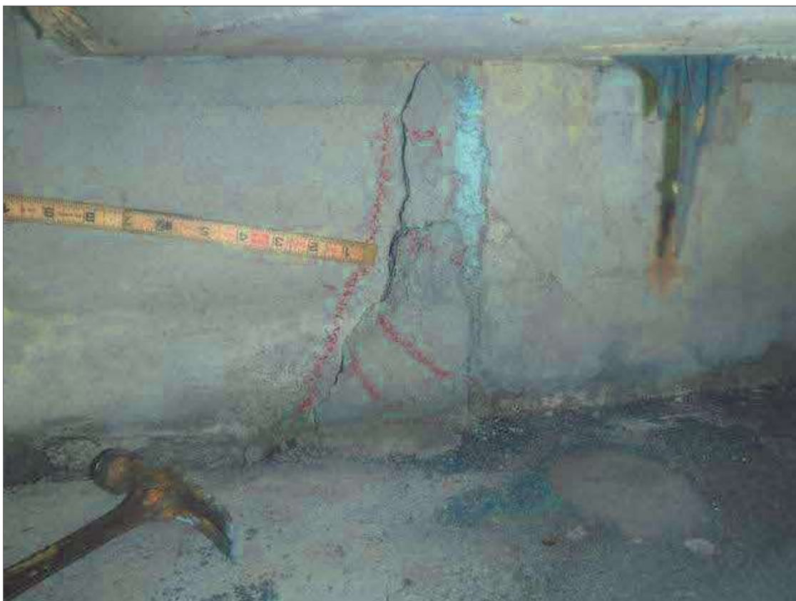
Span 1 Beam 2: 12" X 5" FAILED REPAIR WITH UP TO 1/8" DIAGONAL CRACKS IN RIGHT FACE OF GIRDER AT PIER 1
