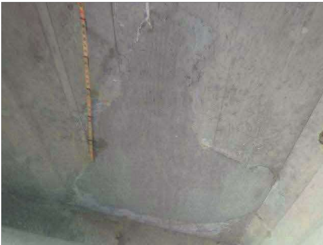
Span 1 Deck: 52" X 43" PATCH IN BOTTOM OF DECK IN BAY 2 NEAR ABUTMENT 1
