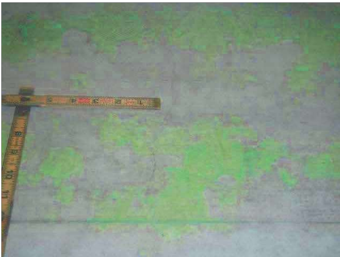
Span 4 Beam 1: UP TO 0.012" TRANSVERSE AND VERTICAL CRACKS IN BOTTOM AND BOTH FACES OF GIRDER IN VARIOUS LOCATIONS THROUGHOUT, CONDITION ON RIGHT SIDE NEAR MIDSPAN SHOWN
