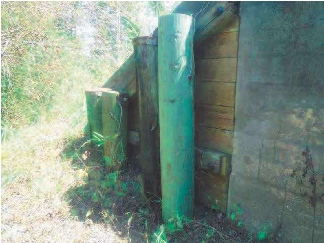
PRIORITY MAINTENANCE REPAIR TO SOUTHWEST WINGWALL BRACE PILE 1 WITH ADDITION OF PILE TO RIGHT OF ORIGINAL PILE SINCE 2018 INSPECTOIN
