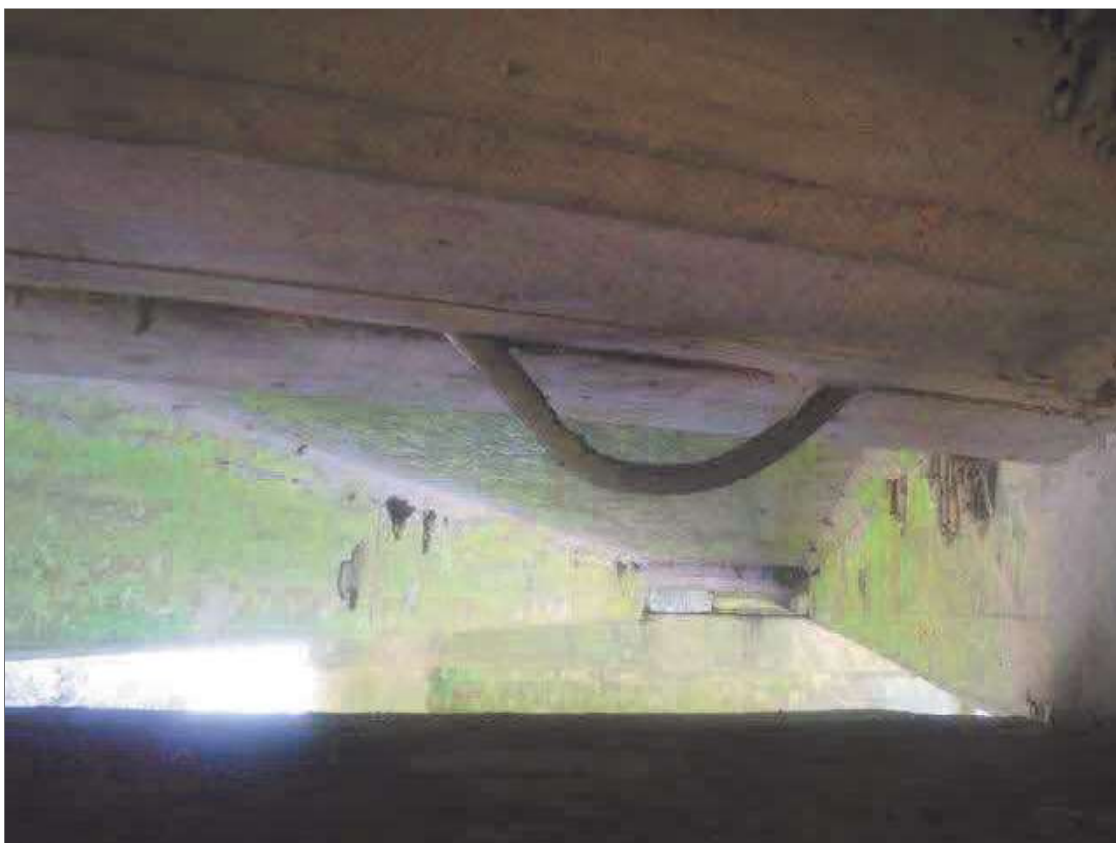
Span 4 Expansion Joint 3: BROKEN AND HANGING BACKER ROD ALONG PIER 3 JOINT IN VARIOUS LOCATIONS THROUGHOUT BAYS, CONDITION IN BAY 2 SHOWN
