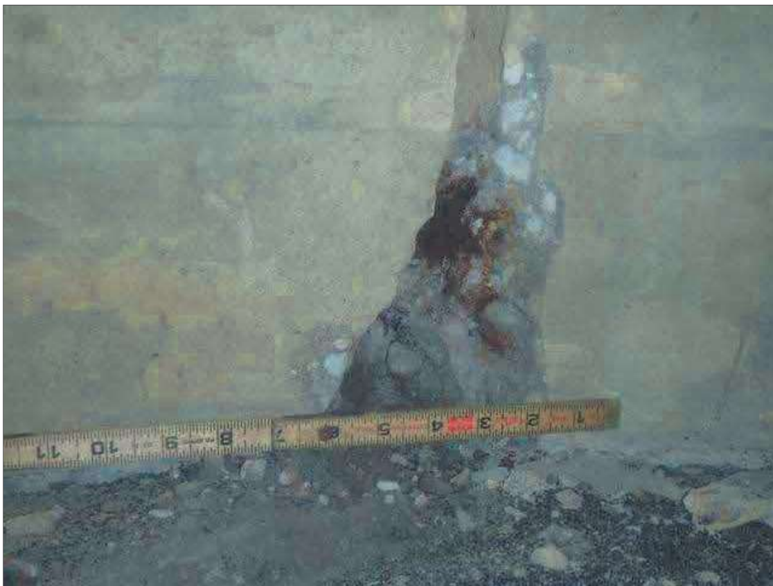
Span 3 Beam 2: PAR: 9" X 2" X 2" DEEP SPALL WITH EXPOSED REBAR IN LEFT FACE OF GIRDER AT PIER 3
