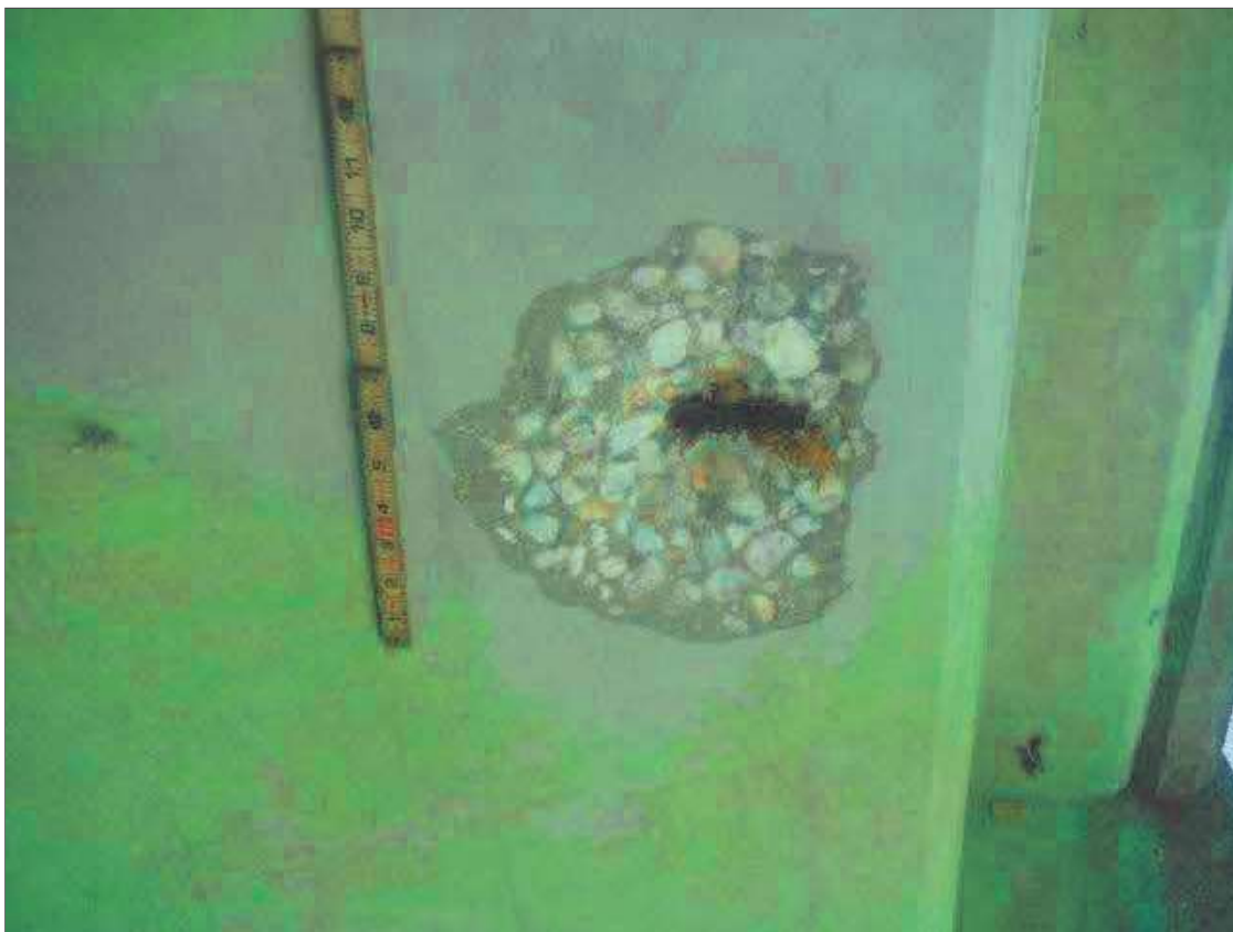
Span 3 Deck: 10" X 8" X 1" DEEP SPALL WITH EXPOSED REBAR IN BOTTOM OF RIGHT OVERHANG NEAR PIER 3
