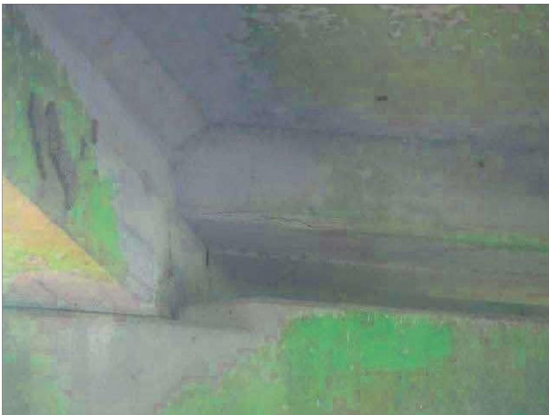
Span 2 Beam 3: UP TO 1/16" HORIZONTAL CRACKS IN FACE OF PIER 1 DIAPHRAGM IN BAY 3, ADJACENT TO GIRDER 4
