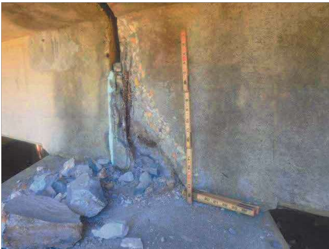
Span 1 Beam 1: PAR: 21" X 10" X 4" DEEP SPALL WITH EXPOSED REBAR IN LEFT FACE OF GIRDER AT PIER 1
