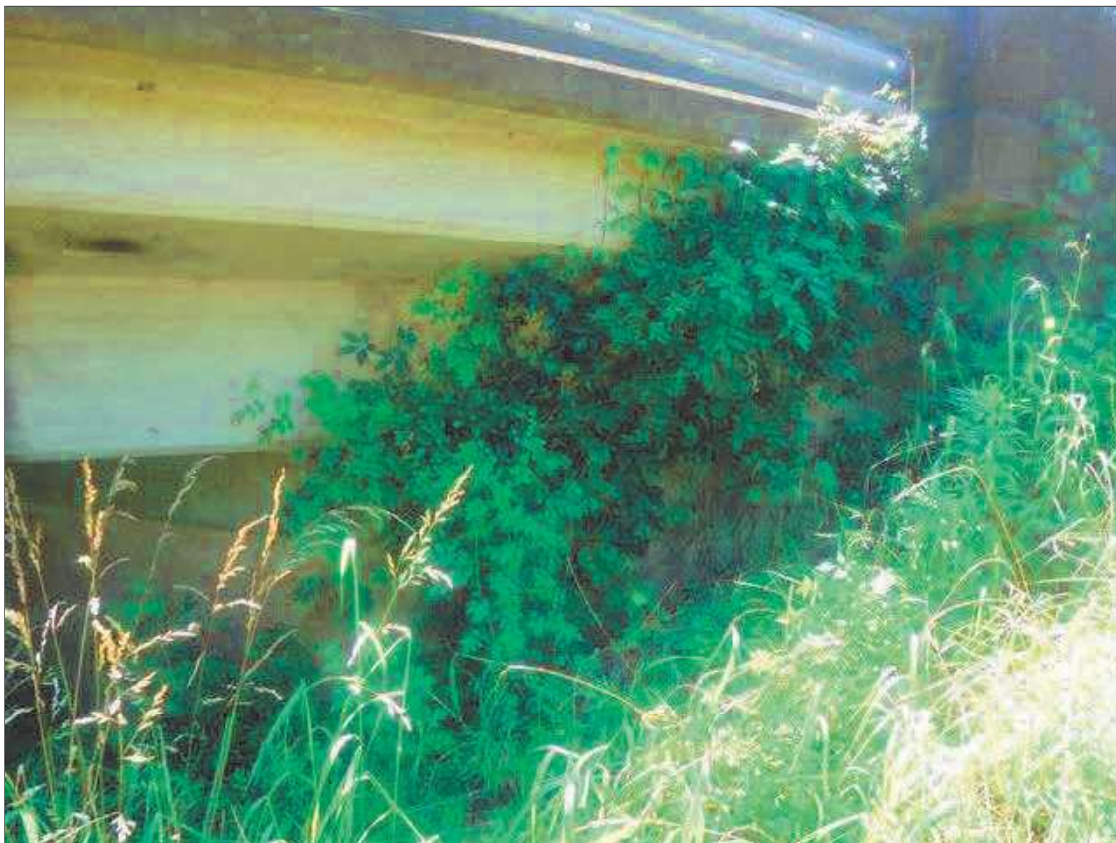
Span 1 Deck: VEGETATION GROWTH ALONG ABUTMENT 1 AT LEFT END, EXTENDING TO BOTTOM OF DECK
