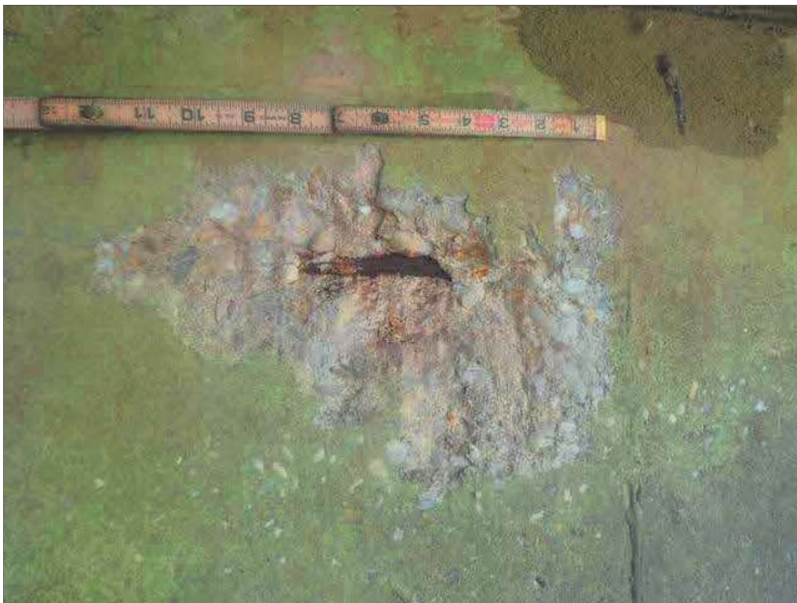
Bent 1 Pile 1: 12" X 6" X 1" DEEP SPALL WITH EXPOSED REBAR IN SPAN 1 FACE OF PIER WALL, APPROXIMATELY 1' FROM BOTTOM OF CAP
