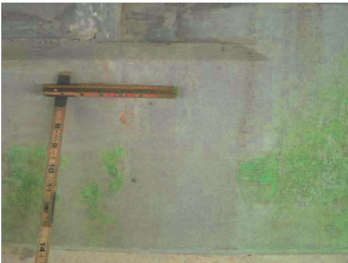
End Bent 1 Cap 1: UP TO 0.012" VERTICAL CRACKS IN FACE OF CAP IN VARIOUS LOCATIONS THROUGHOUT, CRACK IN BAY 2 TO LEFT OF GIRDER 3 SHOWN
