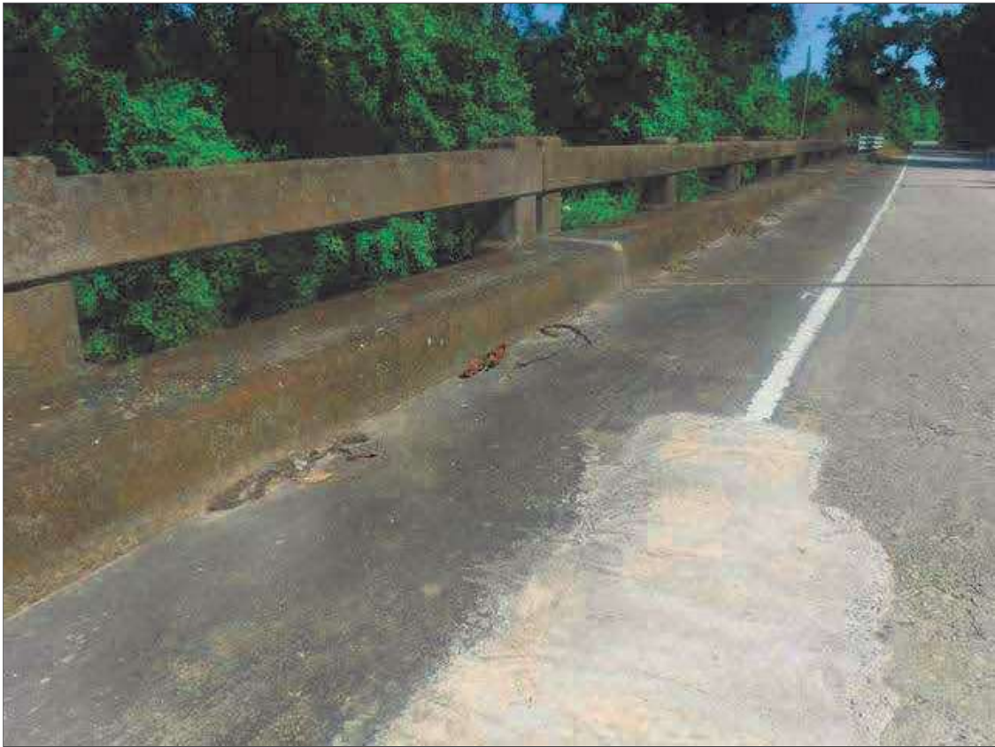
DIRT AND DEBRIS ACCUMULATION IN BOTH SHOULDERS, ACCUMULATION IN LEFT SHOULDER SHOWN
