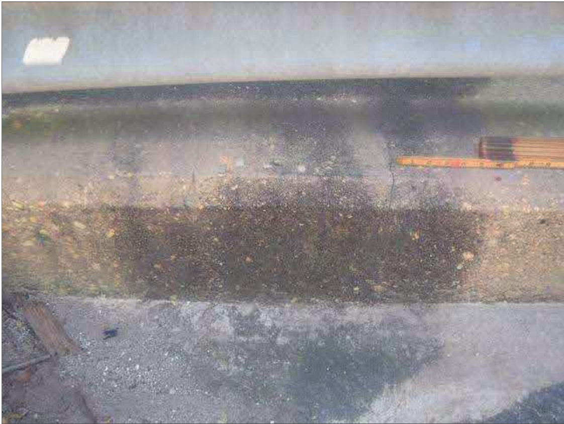
Span 1 Left Bridge Rail: UP TO 0.025" TRANSVERSE AND VERTICAL CRACKS IN TOP AND FACE OF CURB NEAR ABUTMENT 1 FILL FACE
