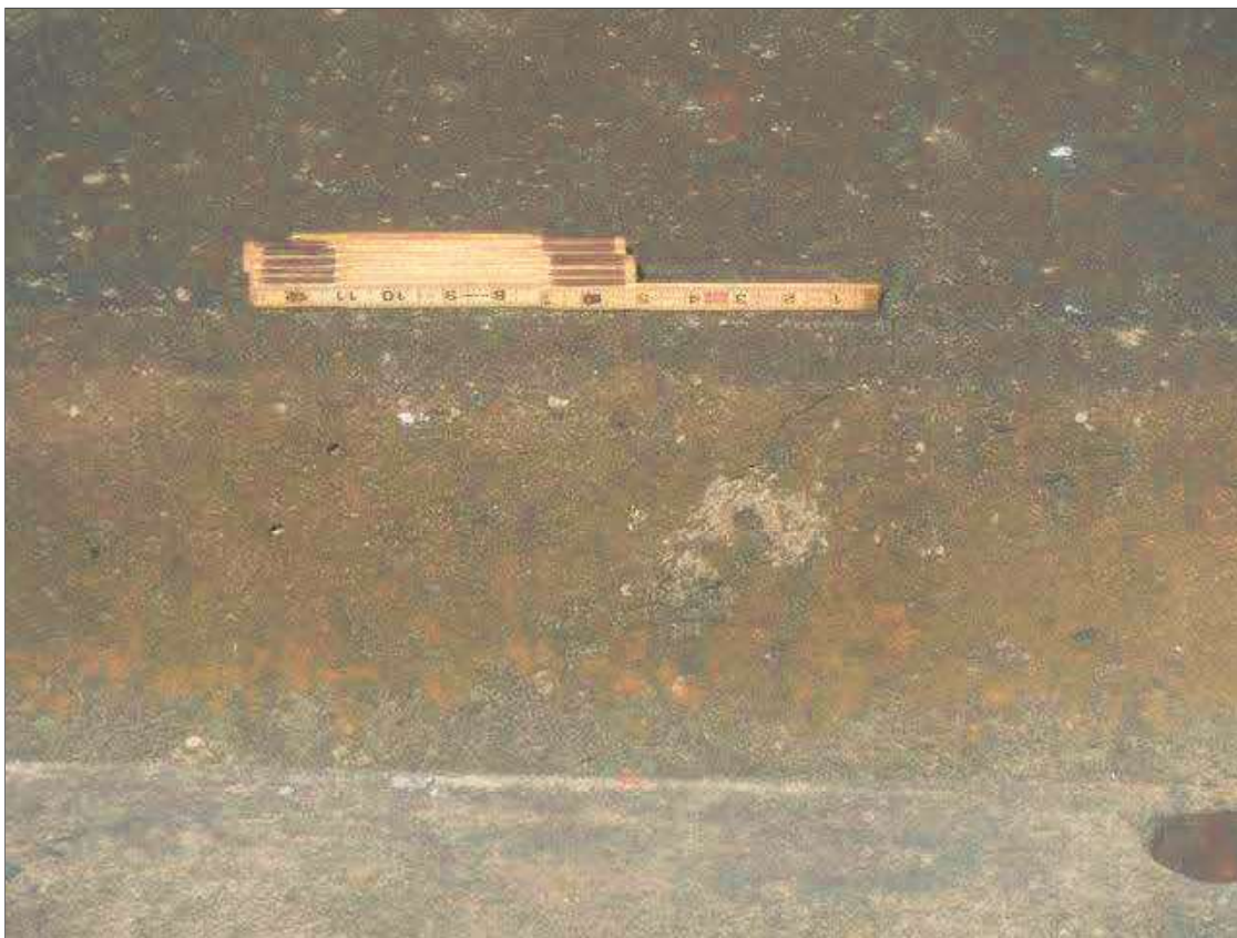
Span 3 Right Bridge Rail: UP TO 1/16" DIAGONAL CRACK IN TOP AND FACE OF CURB, APPROXIMATELY 4' FROM PIER 3 JOINT
