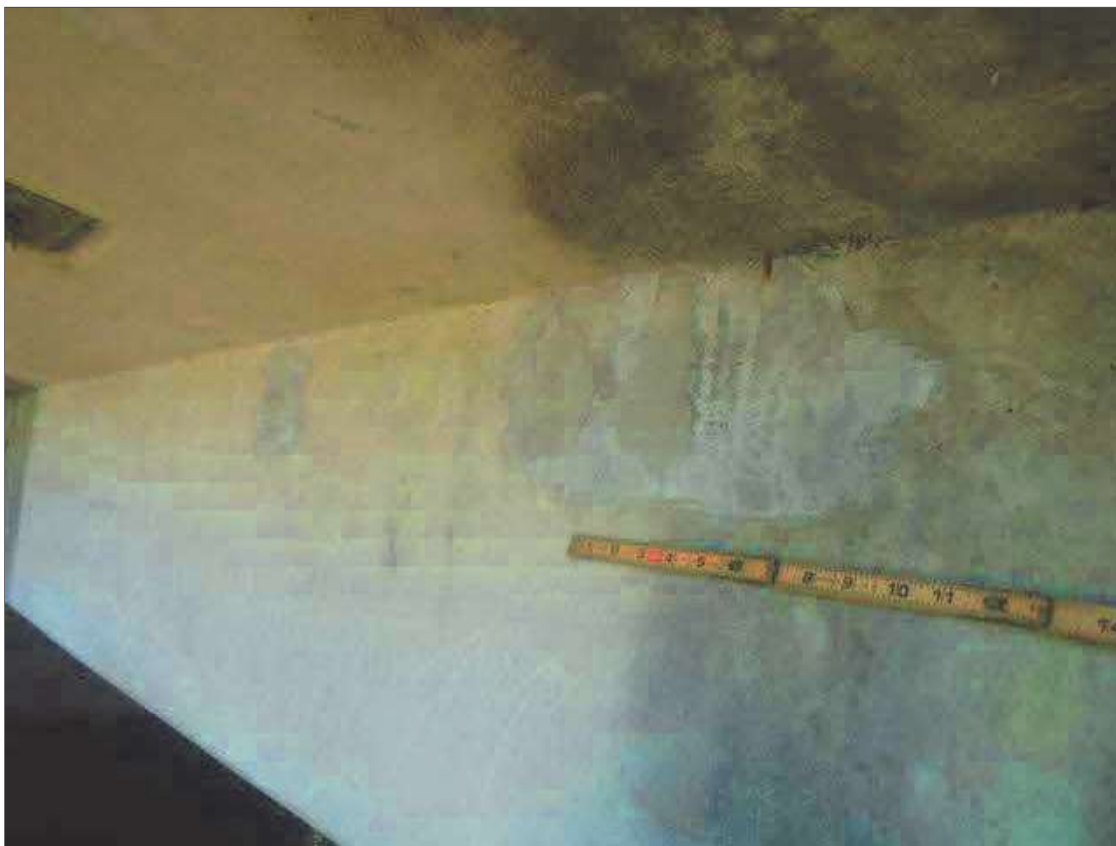
Span 2 Beam 1: (2) REPAIRS UP TO 14" X 6" IN LEFT FACE OF GIRDER, APPROXIMATELY 1' AND 3' FROM PIER 1
