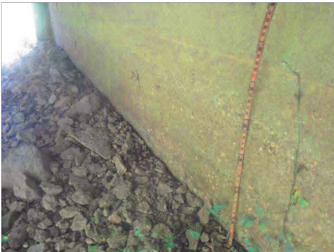
Bent 3 Pile 1: UP TO 38" HIGH SCALING WITH EXPOSED AGGREGATE THROUGHOUT PIER WALL, CONDITION IN SPAN 3 FACE SHOWN
