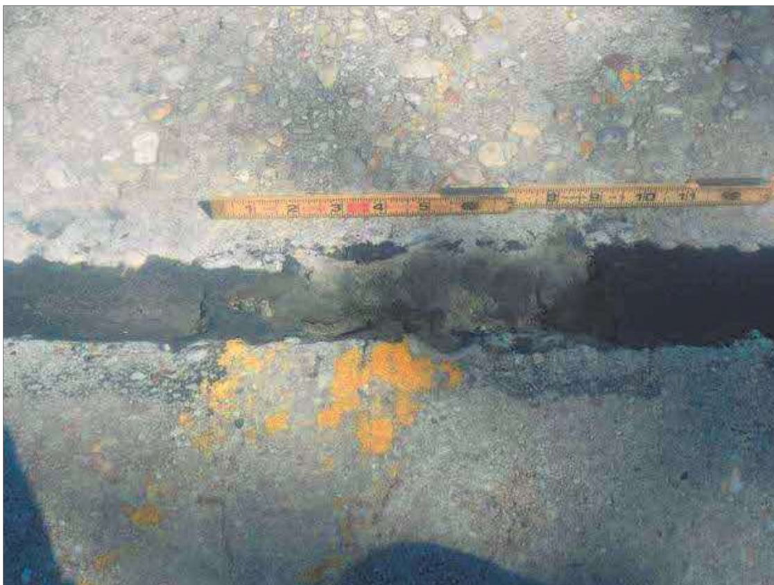
Span 3 Expansion Joint 2: 9" SECTION OF MISSING JOINT MATERIAL ALONG PIER 2 JOINT AT CENTERLINE OF ROADWAY
