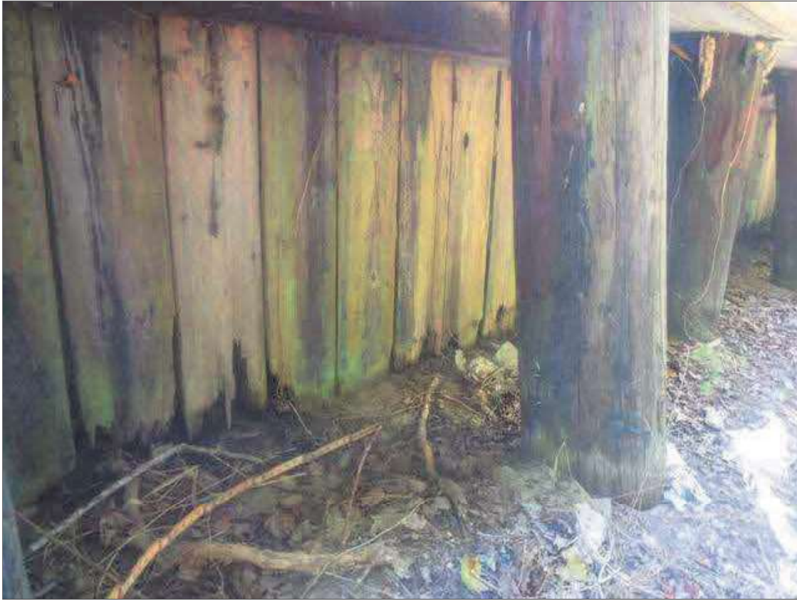
PAR: 50' SECTION WITH AREAS OF DECAY UP TO FULL DEPTH WITH EXPOSED FILL THROUGHOUT FACE OF SOUTHEAST WINGWALL, BEGINNING APPROXIMATELY 18' FROM NEAR END OF WINGWALL, CONDITION APPROXIMATELY 40' FROM NEAR END OF WINGWALL SHOWN
