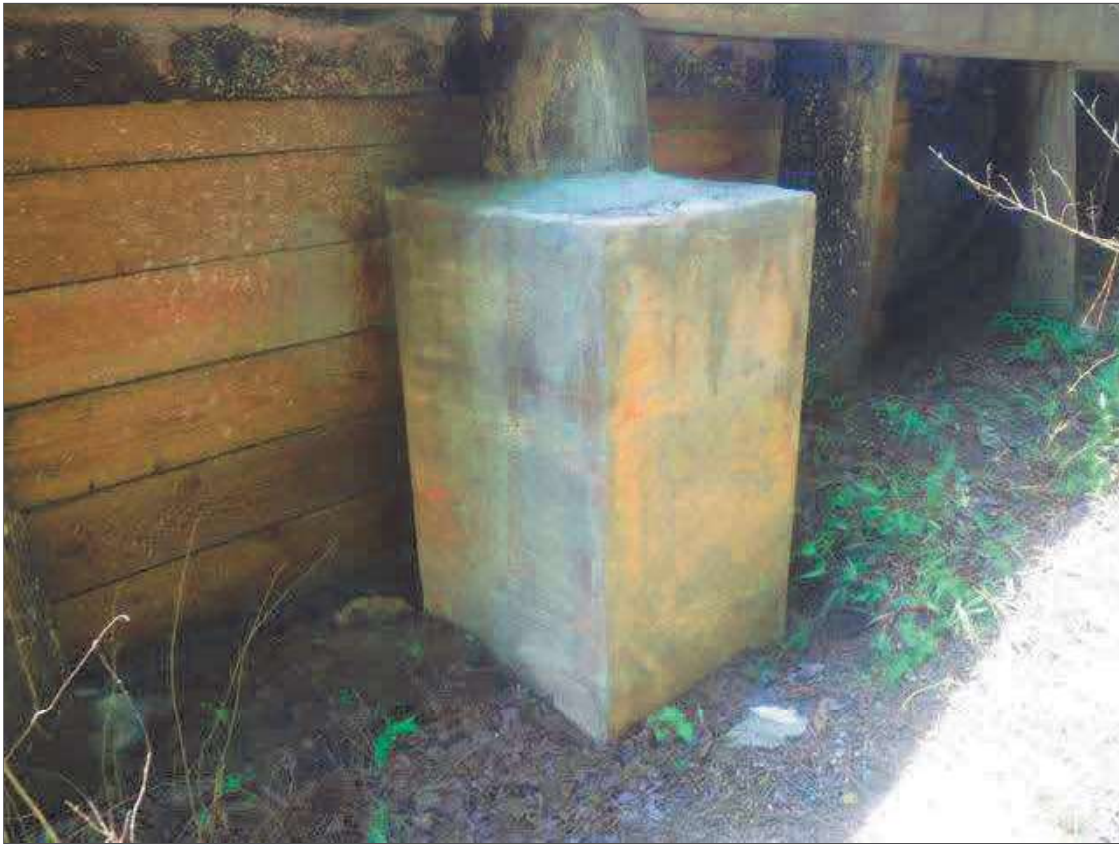
PRIORITY MAINTENANCE REPAIR TO SOUTHEAST WINGWALL BRACE PILE 4 SINCE 2018 INSPECTOIN, APPROXIMATELY 13' FROM NEAR END OF SOUTHEAST WINGWALL
