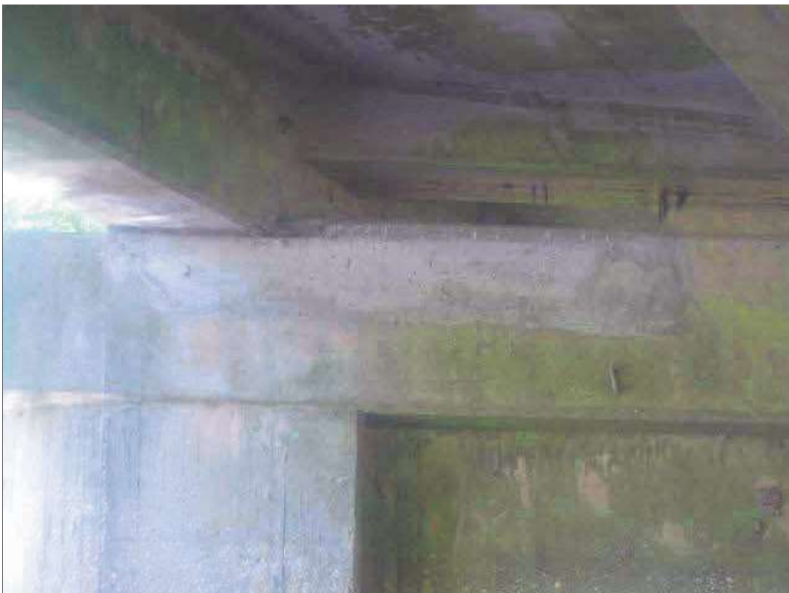
Bent 2 Cap 1: APPROXIMATELY 7' X 12" REPAIR IN SPAN 2 FACE OF CAP BENEATH BAY 1
