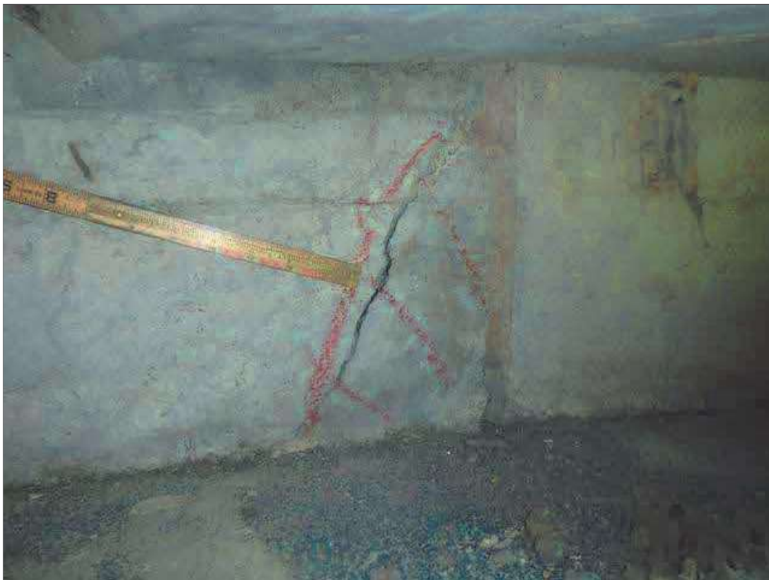
Span 1 Beam 1: 10" X 5" AREA OF DELAMINATION WITH UP TO 1/4" DIAGONAL CRACK IN RIGHT FACE OF GIRDER AT PIER 1
