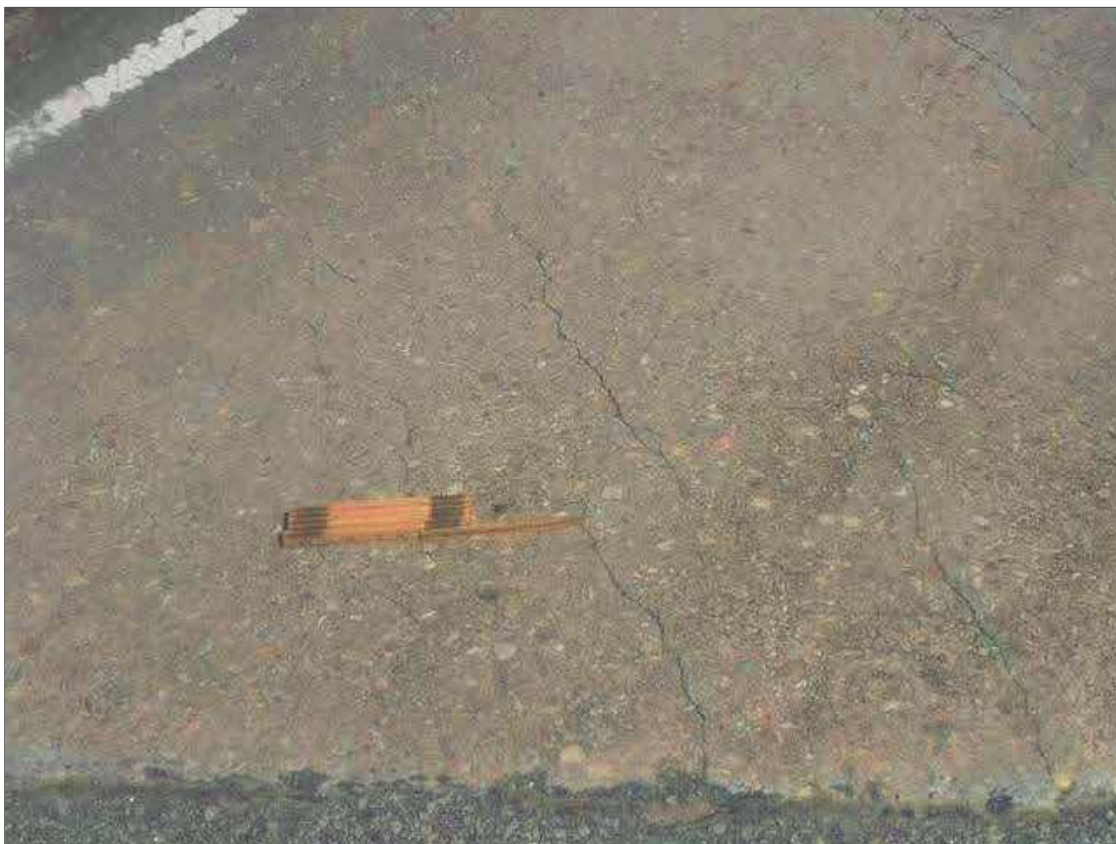
Span 1 Deck: UP TO 1/16" DIAGONAL CRACKS IN TOP OF DECK IN WESTBOUND LANE NEAR ABUTMENT 1 FILL FACE
