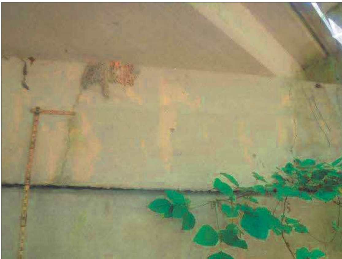
End Bent 2 Abutment: UP TO 0.025" VERTICAL CRACKS IN FACE OF CURTAIN WALL AT RIGHT END
