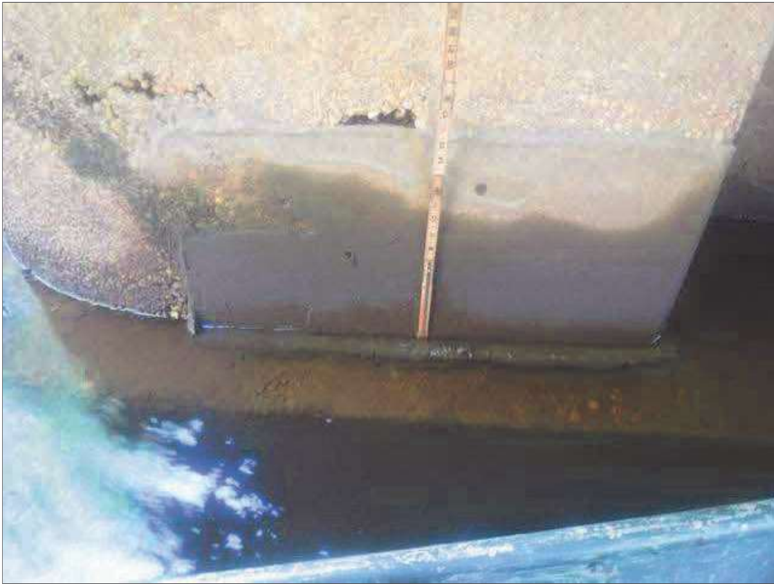
Bent 2 Pile 1: 33" X 16" REPAIR IN SPAN 3 FACE OF PIER WALL AT TOP OF FOOTING BENEATH GIRDER 4
