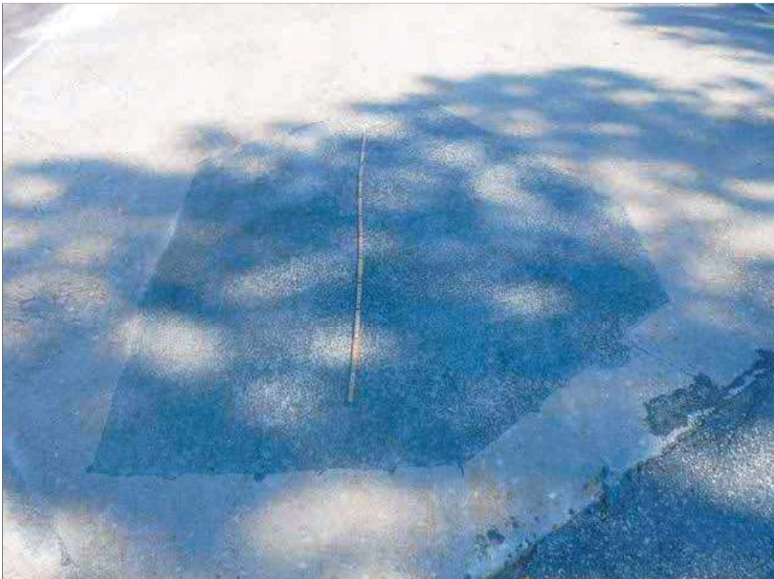
Span 1 Deck: 106" X 77" PATCH IN TOP OF DECK IN CENTERLINE OF ROADWAY NEAR ABUTMENT 1 FILL FACE
