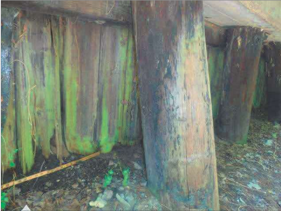
PAR: 50' SECTION WITH AREAS OF DECAY UP TO FULL DEPTH WITH EXPOSED FILL THROUGHOUT FACE OF SOUTHEAST WINGWALL, BEGINNING APPROXIMATELY 18' FROM NEAR END OF WINGWALL, CONDITION APPROXIMATELY 20' FROM NEAR END OF WINGWALL SHOWN
