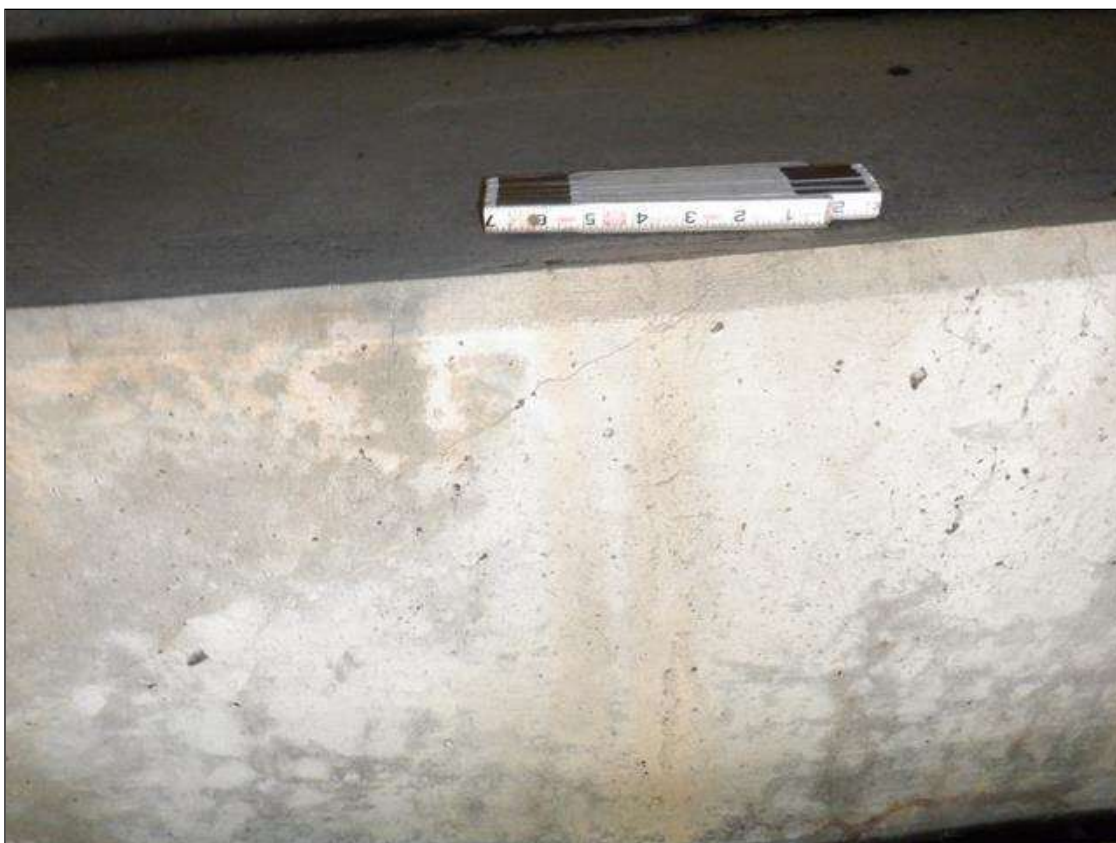
End Bent 1 Cap 1: SCATTERED VERTICAL HAIRLINE CRACKS UP TO 1 FOOT HIGH ALONG FACE OF END BENT CAP
