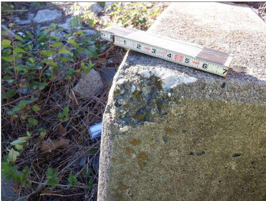
NORTHEAST WINGWALL AT TOP LEFT CORNER, SPALL, 4 INCH DIAMETER X 1/4 INCH DEEP
