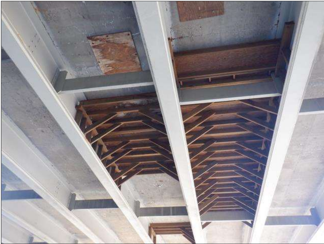
Span 3 Deck: IN BAYS 2 AND 3, SCATTERED FORMWORK LEFT IN PLACE
