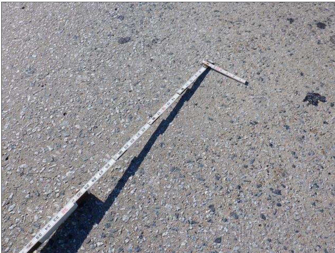
Span 1 Deck: HAIRLINE MAP CRACKING TOPSIDE WITH WEARING SCATTERED THROUGHOUT
