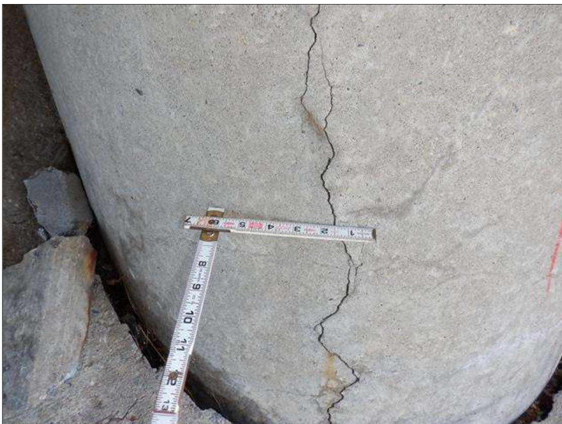
Bent 1 Pile 2: 1/4 INCH VERTICAL CRACKING UP TO 8 FEET HIGH
