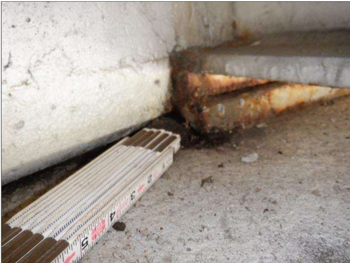
Span 1 Beam 2 - Near Bearing: SURFACE CORROSION ON BEARING PLATES
