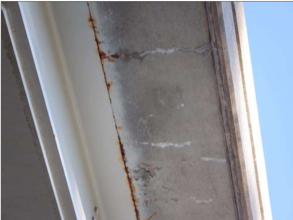
Span 3 Deck: SCATTERED THROUGHOUT BOTH OVERHANGS, HAIRLINE TRANSVERSE CRACKS WITH EFFLORESCENCE
