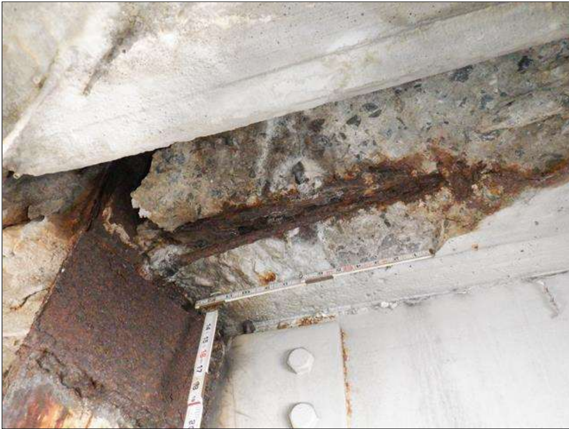
Span 3 Deck: PAR: 2 FEET X 10 INCH X 5 INCH DEEP SPALL WITH EXPOSED REBAR, 5 PERCENT SECTION LOSS, IN UNDERSIDE OF BAY 5 OVER BENT 2
