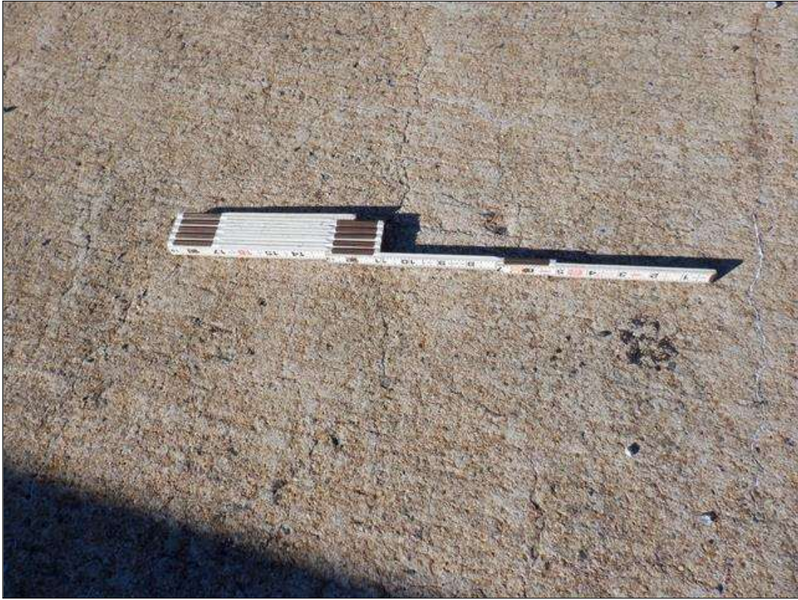
Span 2 Deck: HAIRLINE MAP CRACKING IN TOP OF LEFT AND RIGHT SHOULDERS FOR FULL WIDTH OF SHOULDER X FULL LENGTH OF SPAN
