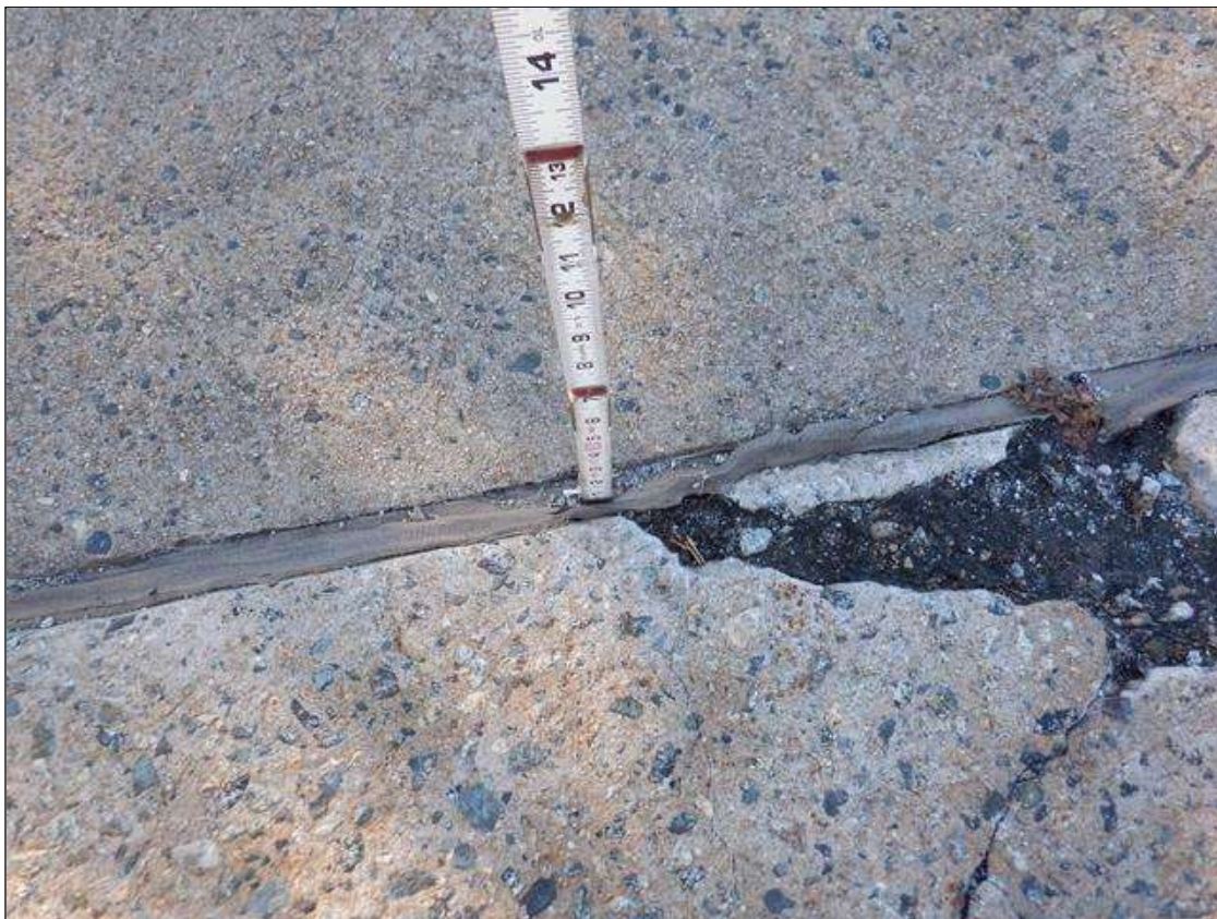
Span 4 Expansion Joint: LOSS OF SEAL ADHESION ALONG EXPOSED JOINT IN SHOULDERS
