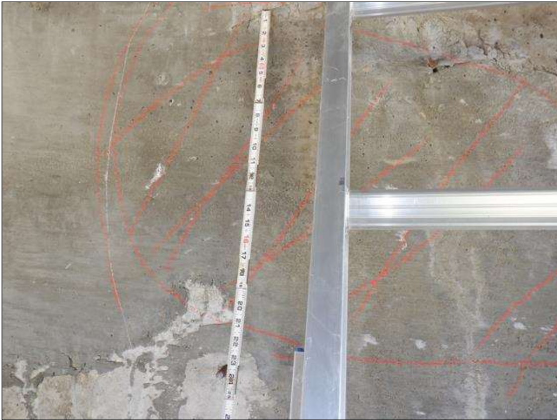
Bent 2 Cap 1: PATCHED PREVIOUS PRIORITY MAINTENANCE ON WEST FACE UNDER GIRDER 5 WITH DELAMINATED AREAS UP TO 2 FOOT DIAMETER
