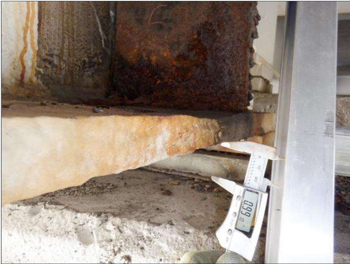
Span 3 Beam 2: CORROSION WITH SECTION LOSS (0.99 INCH REMAINING) ON BOTH BOTTOM FLANGES FOR OUTER 2 INCH FOR 1 FOOT AT BENT 3
