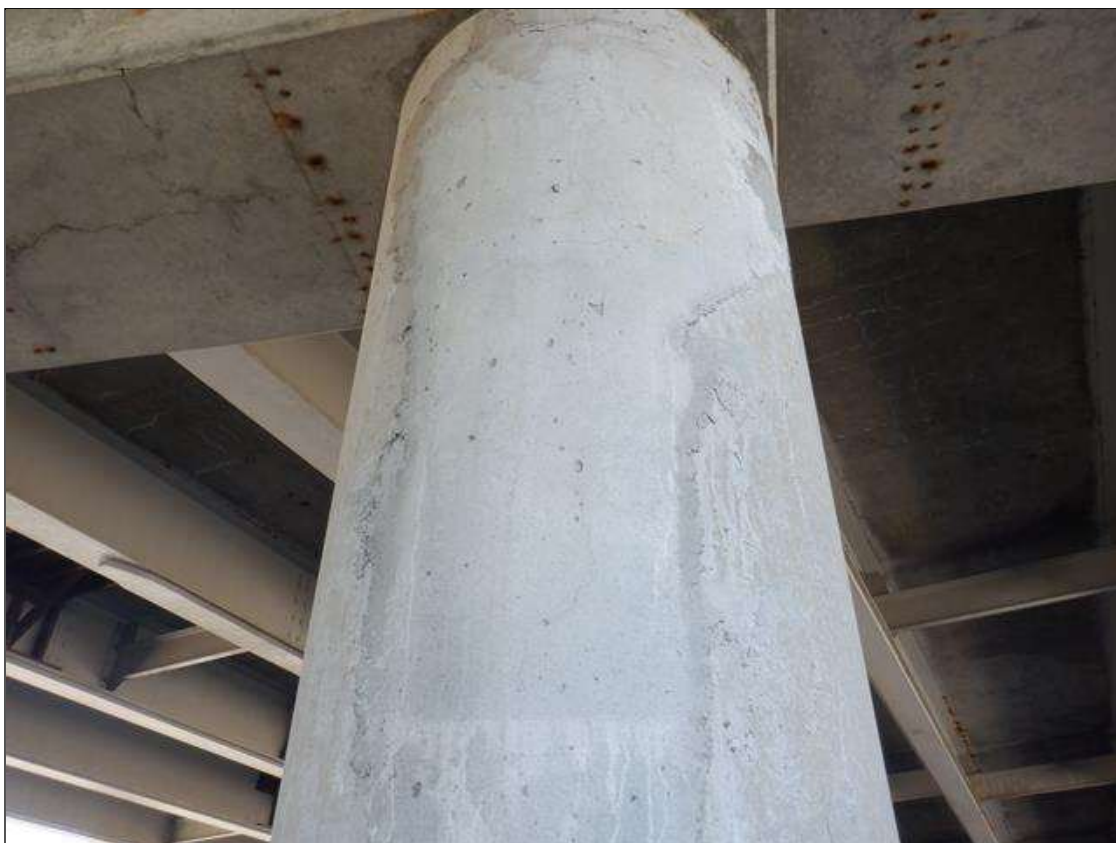
Bent 2 Pile 3: PATCHED AREAS WITH HAIRLINE CRACKS ON WEST FACE AND SOUTH FACE, 4 FEET WIDE X 7 FEET HIGH
