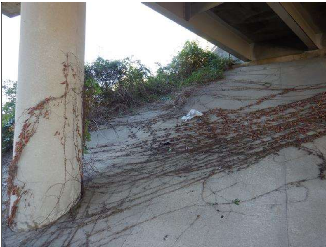
END BENT 1 SLOPE PROTECTION AT PILE 4, 250 SQUARE FEET OF VEGETATION GROWTH
