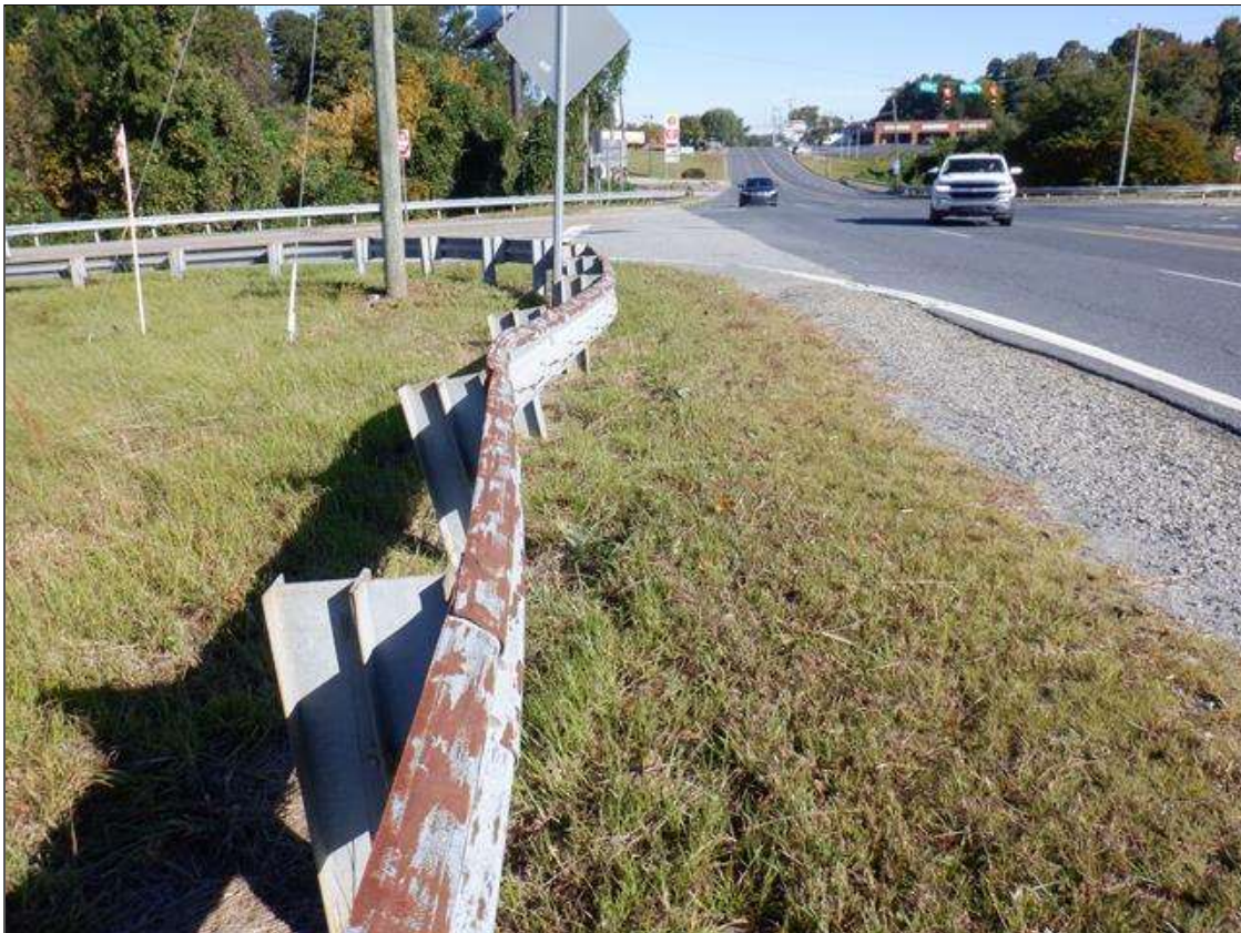
SOUTHWEST GUARDRAIL, STARTING 115 FEET FROM BRIDGE, 20 FEET OF GUARDRAIL DAMAGE WITH UP TO 1 FOOT HORIZONTAL DISPLACEMENT
