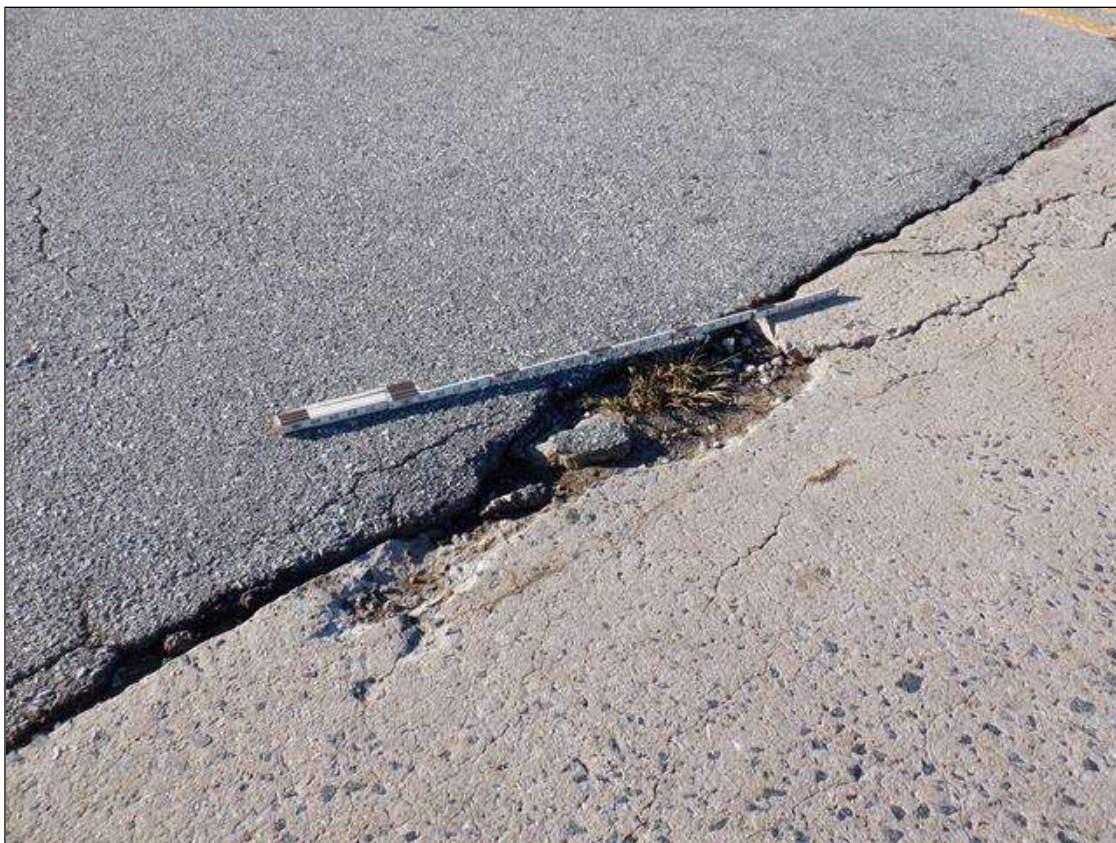
Span 4 Deck: 26 FEET X 3 FEET DELAMINATION AT CENTERLINE AND WESTBOUND LANES AT END BENT 2 WITH (2) SPALLS UP TO 2 FEET X 9 INCH X 1 1/2 INCH DEEP, NO EXPOSED REINFORCEMENT
