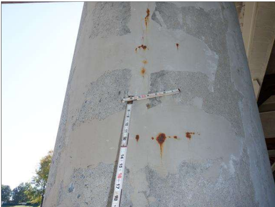
Bent 2 Pile 1: FULL HEIGHT PATCHED AREAS ON WEST FACE WITH RUST STAINS
