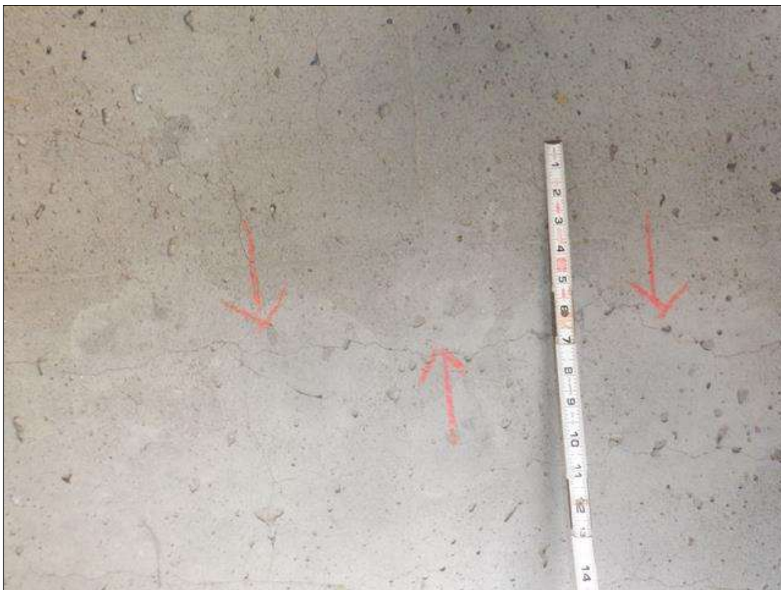
End Bent 1 Abutment: HAIRLINE MAP CRACKING THROUGHOUT FULL LENGTH OF BACKWALL
