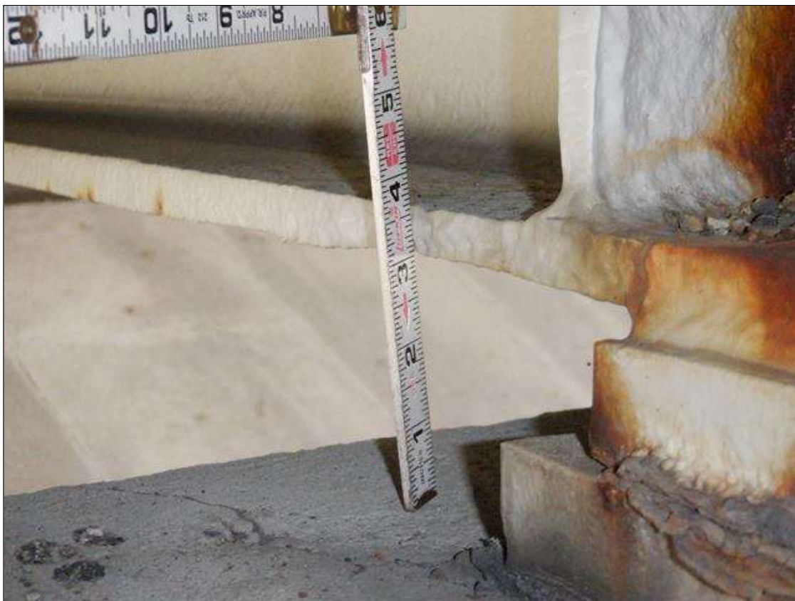
Span 4 Beam 4: CORROSION HAS BEEN ARRESTED WITH PAINT, 3/4 INCH SECTION LOSS (1/2 INCH REMAINING) ON BOTTOM LEFT FLANGE FOR OUTER 2 INCH FOR 18 INCH LONG STARTING 8 INCH FROM BENT 3
