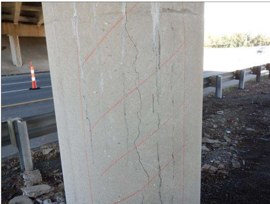
Bent 2 Pile 3: SOUTHEAST FACE STARTING AT GROUND LINE, 6 FOOT HIGH X 2 FOOT WIDE DELAMINATION WITH CRACK UP TO 1/8 INCH WIDE
