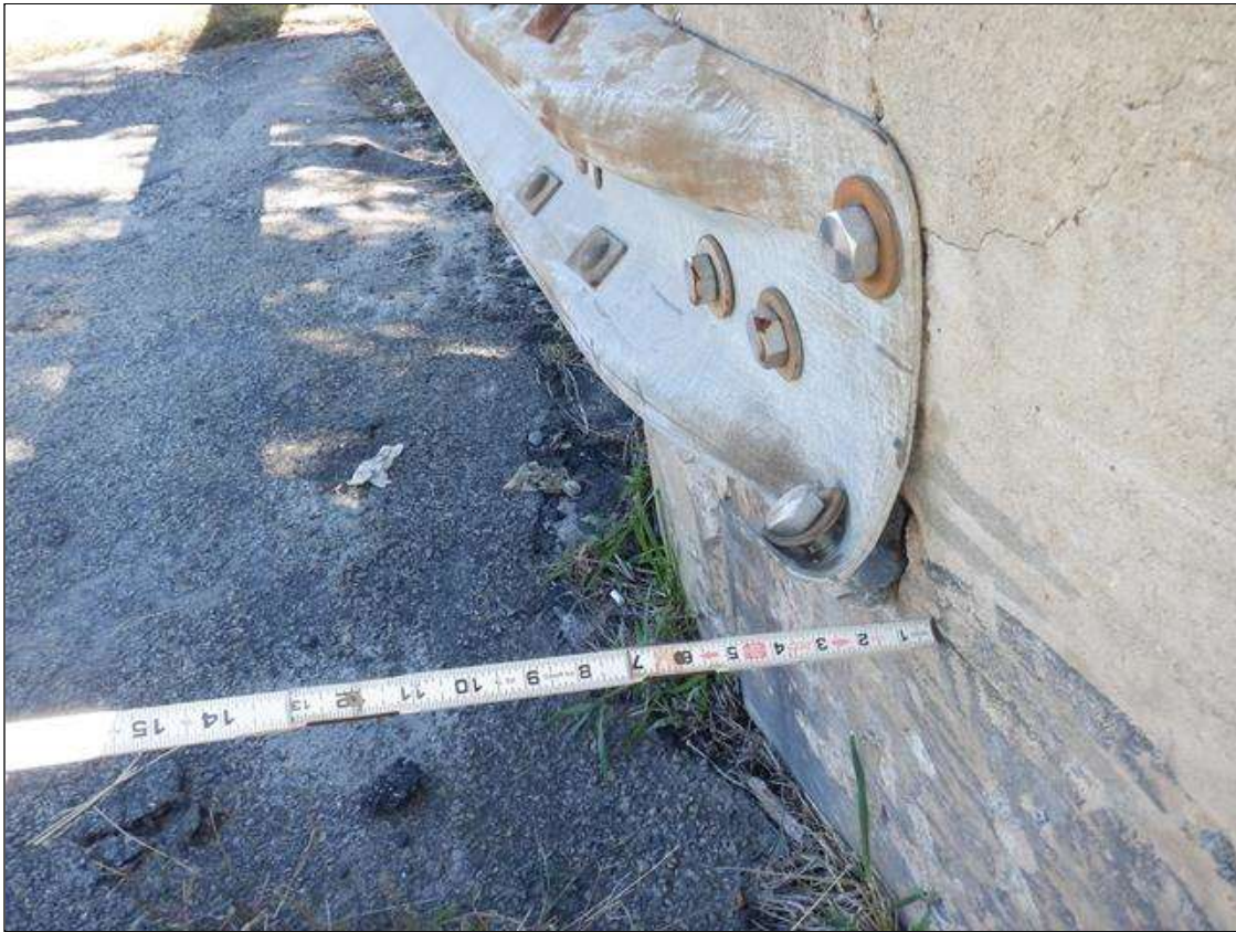
Span 1 Left Bridge Rail: PAR: 1 BOLT OF LEFT GUARDRAIL CONNECTION AT END BENT 1 HAS FAILED, CONNECTION STILL FUNCTIONING
