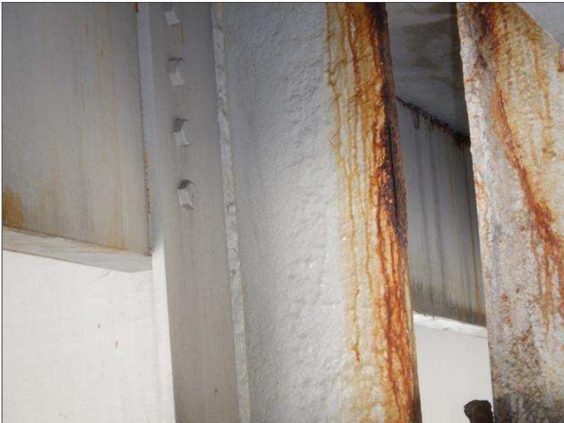
Span 3 Beam 6: CORROSION WITH 1/16 INCH PITTING (11/16 INCH REMAINING) ON FULL HEIGHT OF WEB AT BENT 2
