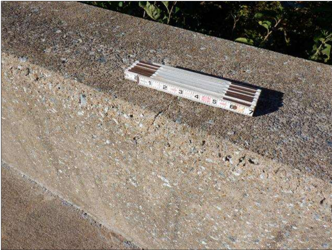
Span 4 Right Bridge Rail: SCATTERED HAIRLINE VERTICAL CRACKING THROUGHOUT, UP TO FULL HEIGHT
