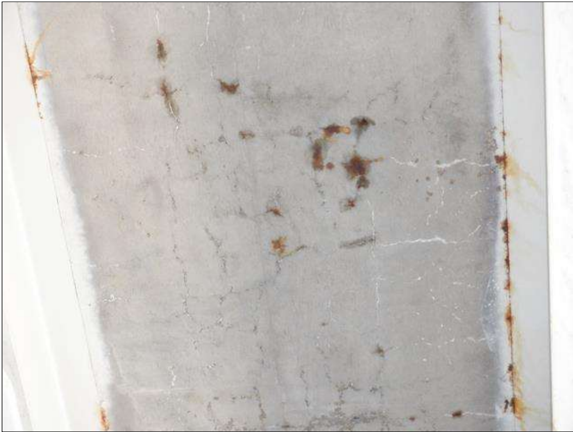
Span 2 Deck: BAY 4 STARTING 15 FEET FROM BENT 2, 2 AREAS UP TO 20 SQUARE FEET OF CRACKING UP TO 1/16 INCH WIDE WITH RUST STAINING
