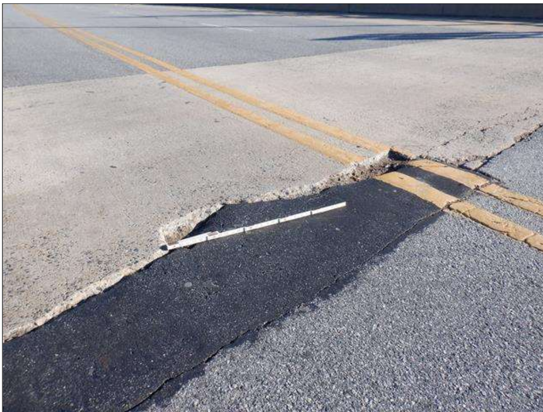
Span 4 Deck: NEAR CENTERLINE OF ROAD IN EASTBOUND LANE, UNSOUND ASPHALT PATCH, 5 FEET WIDE X 2 FEET LONG WITH AREAS OF SPALLS UP TO 2 INCH DEEP
