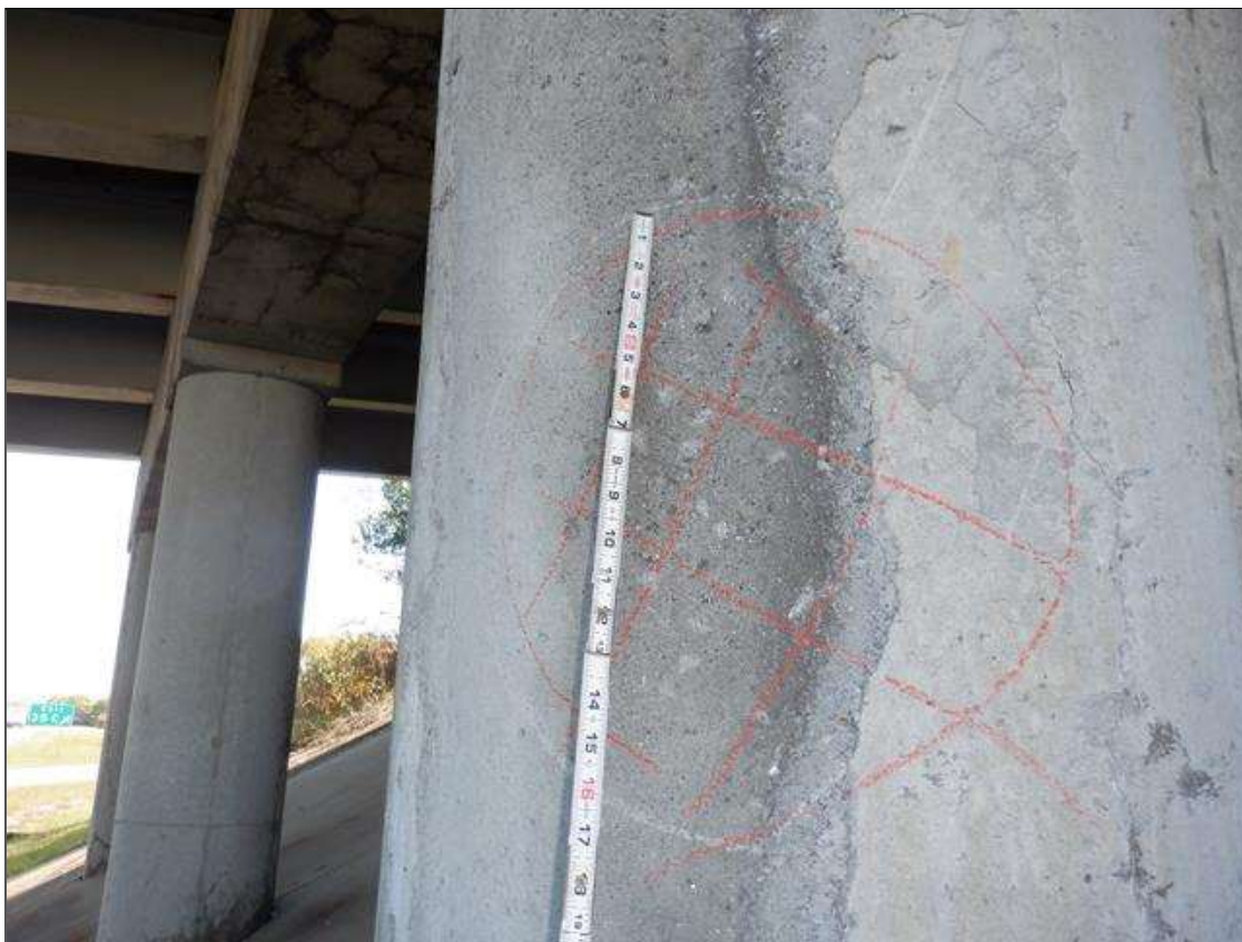
Bent 3 Pile 3: PATCHED AREA, WEST FACE, 2 FEET WIDE X FULL HEIGHT WITH AREA OF DELAMINATION 4 FEET ABOVE GROUND, 16 INCH IN DIAMETER
