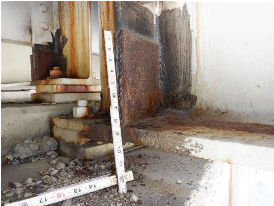
Span 3 Beam 3: WELDED REPAIR TO BOTH SIDES OF BOTH BEARING STIFFENERS AT BENT 3, 9 INCH X 8 INCH X 3/8 INCH THICK STEEL PLATE
