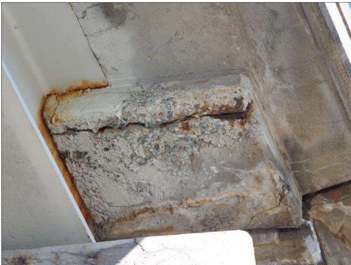
Span 3 Beam 1: PAR: AT BENT 2 LEFT OVERHANG DIAPHRAGM, SPALL 2 FOOT WIDE X 8 INCH LONG X 2 INCH DEEP WITH EXPOSED REBAR, 5 PERCENT SECTION LOSS
