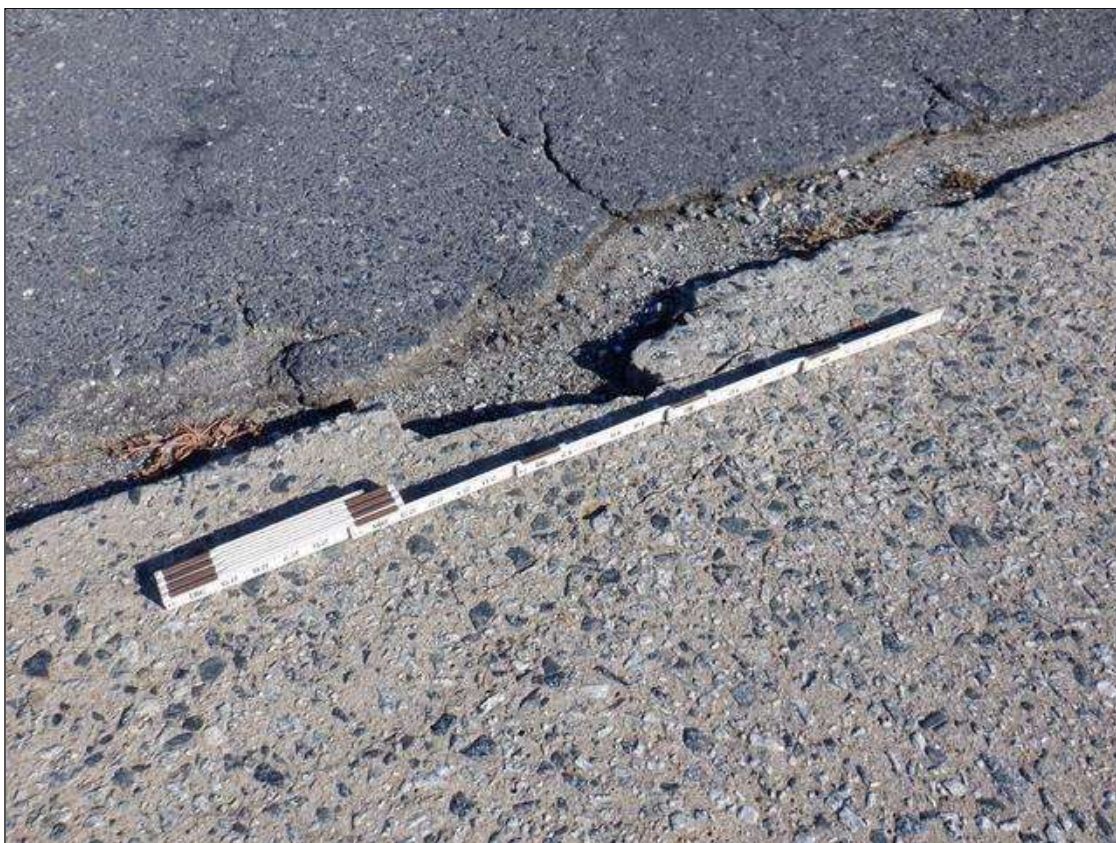
Span 1 Deck: LEFT EASTBOUND LANE, SPALL, 1 FOOT WIDE X 4 INCH LONG X 1 1/2 DEEP
