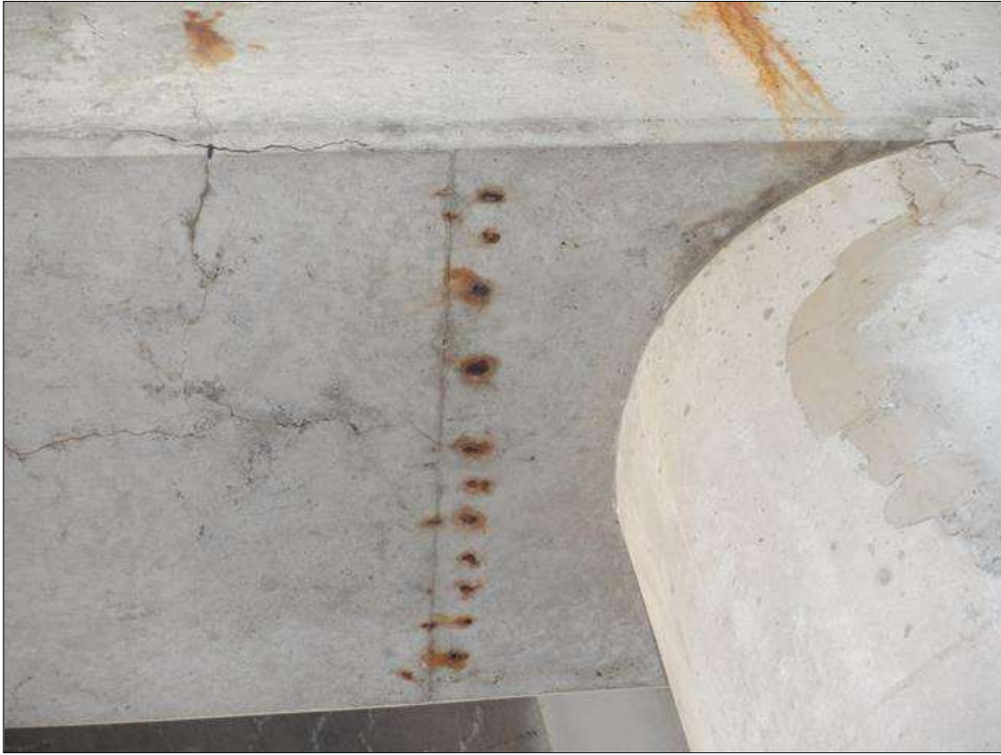
Bent 2 Cap 1: ALONG CAP SOFFIT, 12 FEET OF EXPOSED REBAR CHAIRS
