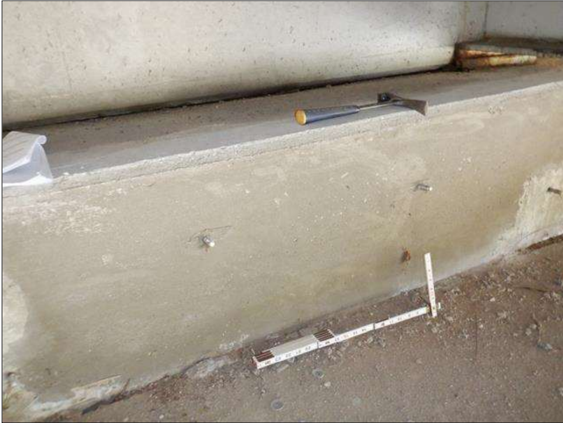
End Bent 1 Cap 1: SOUND PATCHED AREA UNDER BAY 2 AND GIRDER 2, 10 FEET LONG X FULL HEIGHT OF CAP
