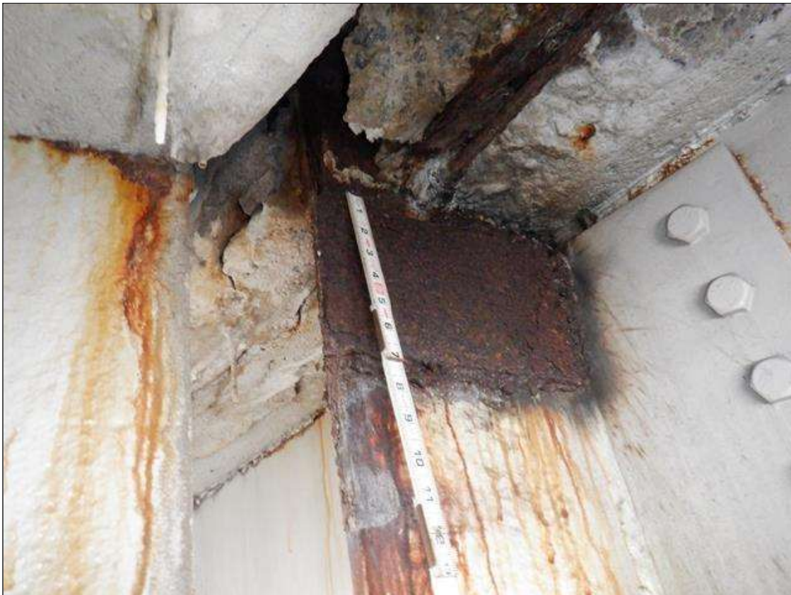
Span 3 Beam 5: AT BENT 2, TOP 6 INCHES OF WEB HAS A REPAIR PLATE, 6 INCH X 6 INCH X 1/2 INCH THICK WITH RUST SCALE
