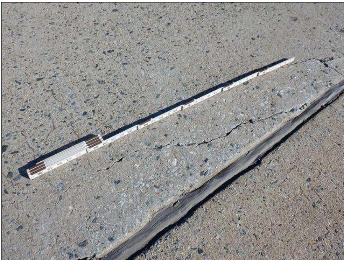
Span 1 Deck: TOP OF DECK IN FAR RIGHT EASTBOUND LANE AT BENT 1, 6 FEET X 1 FOOT DELAMINATION WITH CRACKING UP TO 1/8 INCH WIDE
