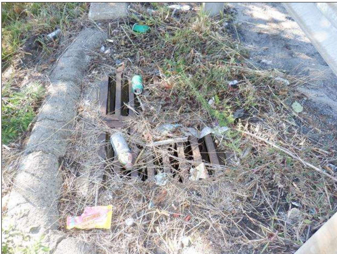
NORTHWEST CATCH BASIN CLOGGED WITH DEBRIS
