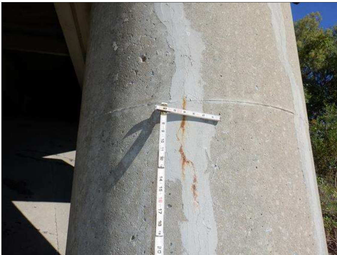
Bent 1 Pile 1: 15 FEET OF SEALED CRACK, SOME WITH RUST STAINING
