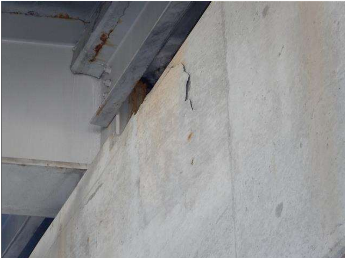
Bent 2 Cap 1: (5) DELAMINATIONS UP TO 1 FOOT DIAMETER SCATTERED THROUGHOUT EAST FACE
