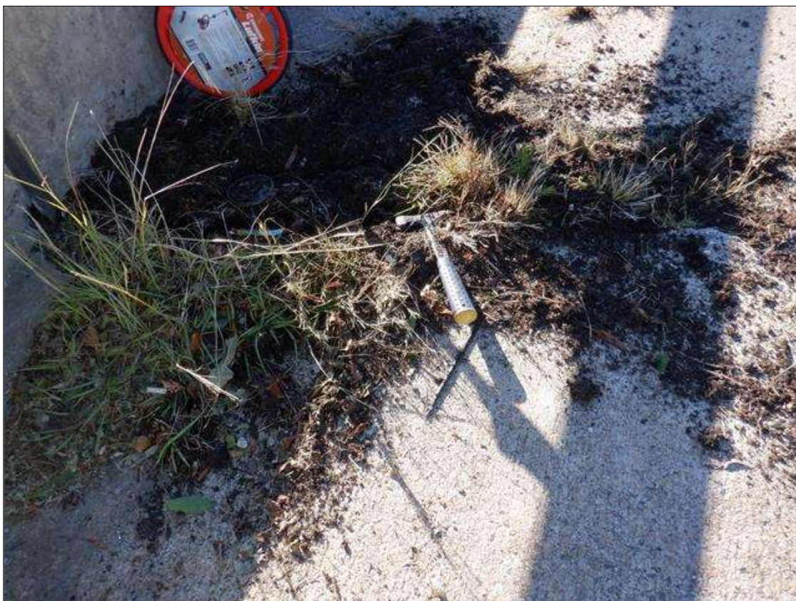
Span 2 Deck: 6 FEET X 6 INCH X 5 INCH DEEP SPALL ON LEFT SHOULDER AT BENT 2 JOINT, REBAR COVERED BY PACKED DEBRIS
