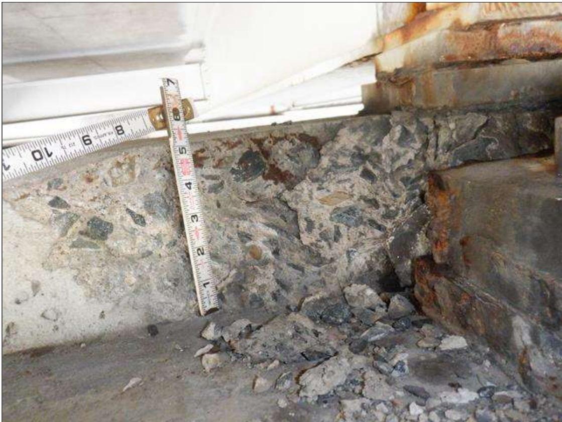
Bent 3 Cap 1: 18 INCH X 6 INCH X 5 INCH SPALL ON PEDESTAL UNDER END OF SPAN 4 GIRDER 4, NO EXPOSED REBAR, NO BEARING LOSS
