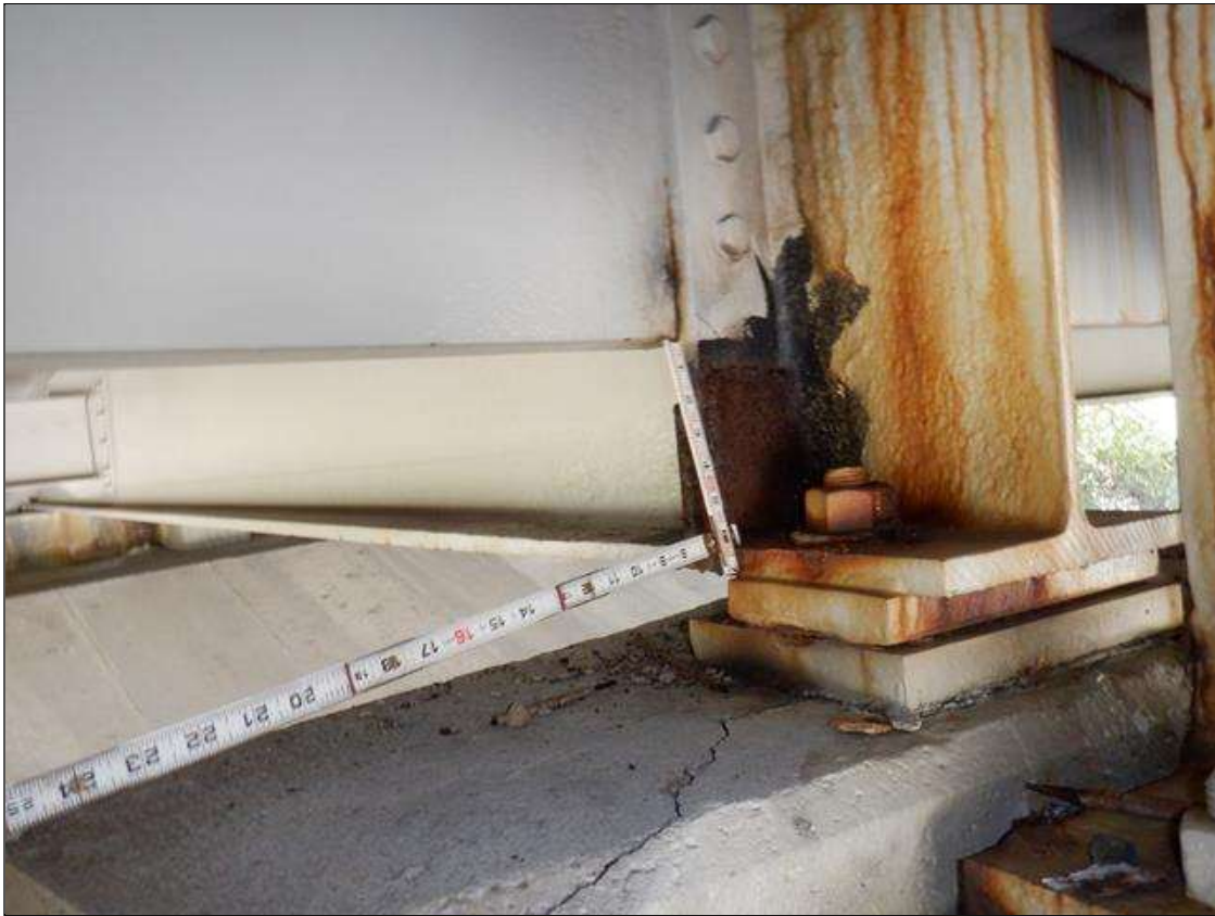
Span 4 Beam 3: AT BENT 3, LEFT BEARING STIFFENER HAS WELDED REPAIR PLATE, 5 INCH X 5 INCH X 1/2 INCH THICK WITH RUST SCALE
