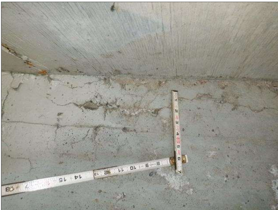
End Bent 2 Abutment: SCATTERED HAIRLINE MAP CRACKING IN BACKWALL OF BAY 3 AND BAY 4, FULL WIDTH X UP TO 2 FEET HIGH
