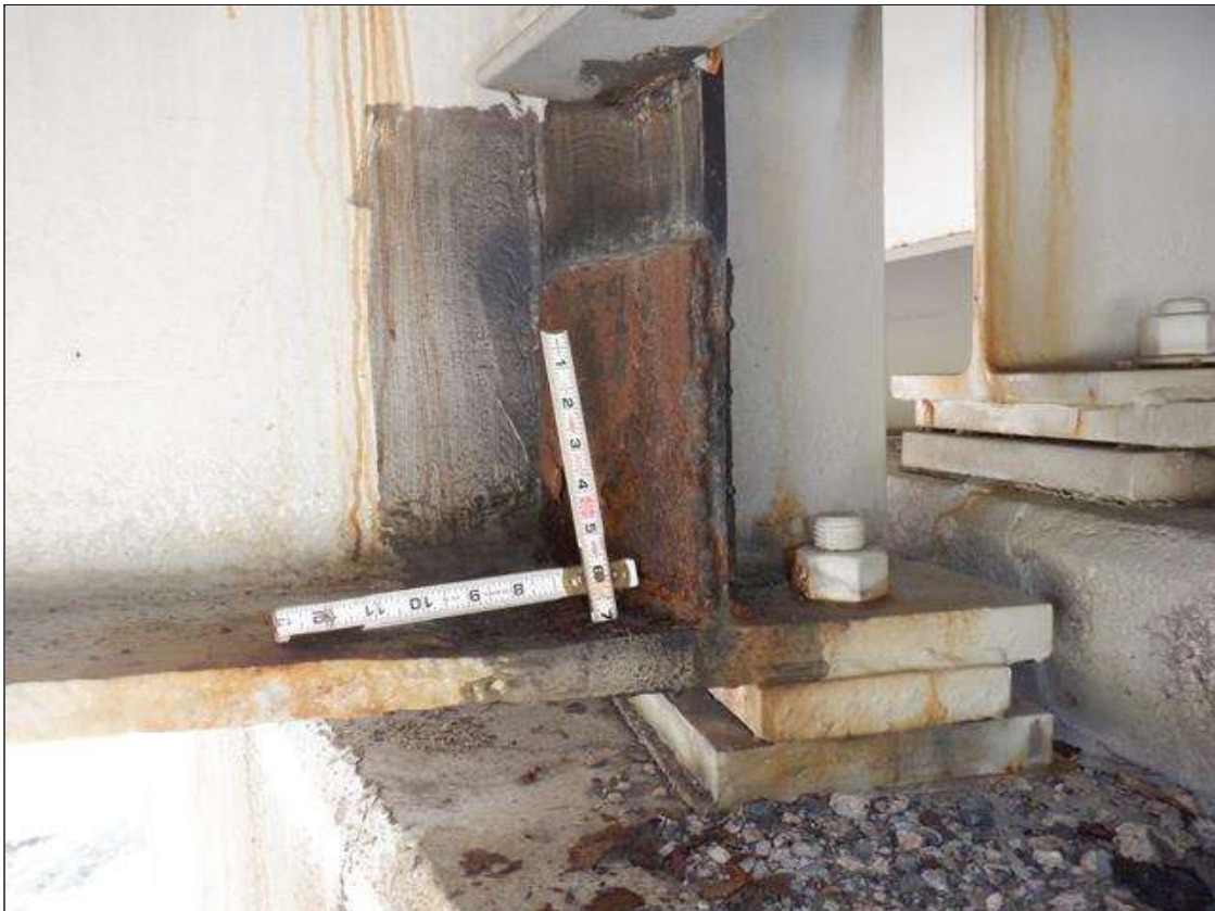
Span 3 Beam 2: WELDED REPAIR TO BOTH SIDES OF BOTH BEARING STIFFENERS AT BENT 3, 9 INCH X 8 INCH X 3/8 INCH THICK STEEL PLATE
