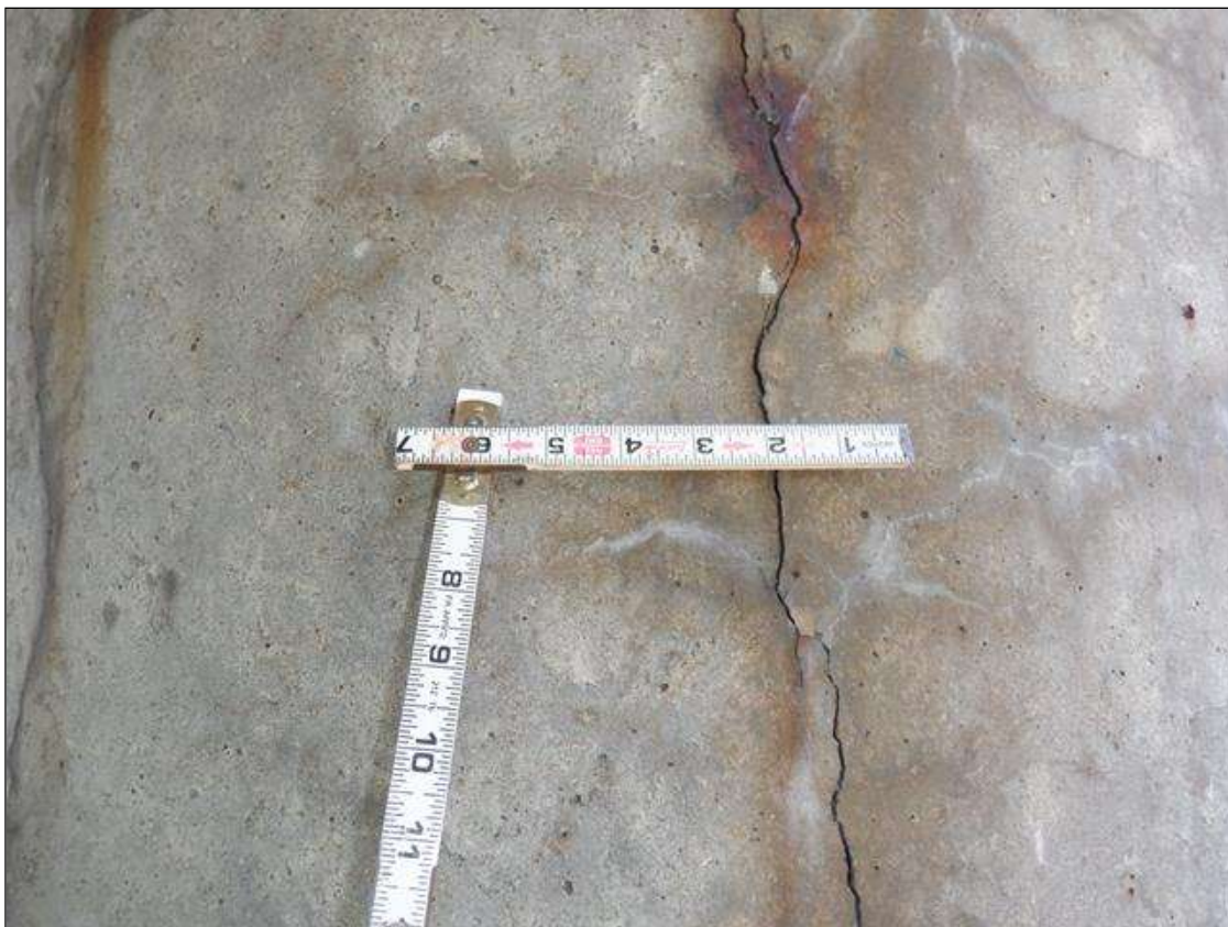
Bent 3 Pile 1: FULL HEIGHT 1/8 INCH WIDE VERTICAL CRACK
