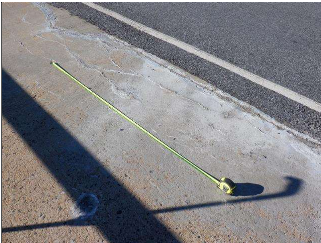
Span 3 Deck: LEFT SHOULDER, UP TO 50 SQUARE FEET OF UNSOUND PATCHED AREAS WITH CRACKS UP TO 1/16 INCH WIDE WITH EFFLORESCENCE
