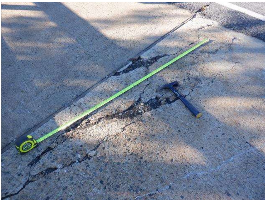
Span 3 Deck: DELAMINATION 360 SQUARE FEET IN WESTBOUND SHOULDER AND 360 SQUARE FEET IN EASTBOUND SHOULDER
