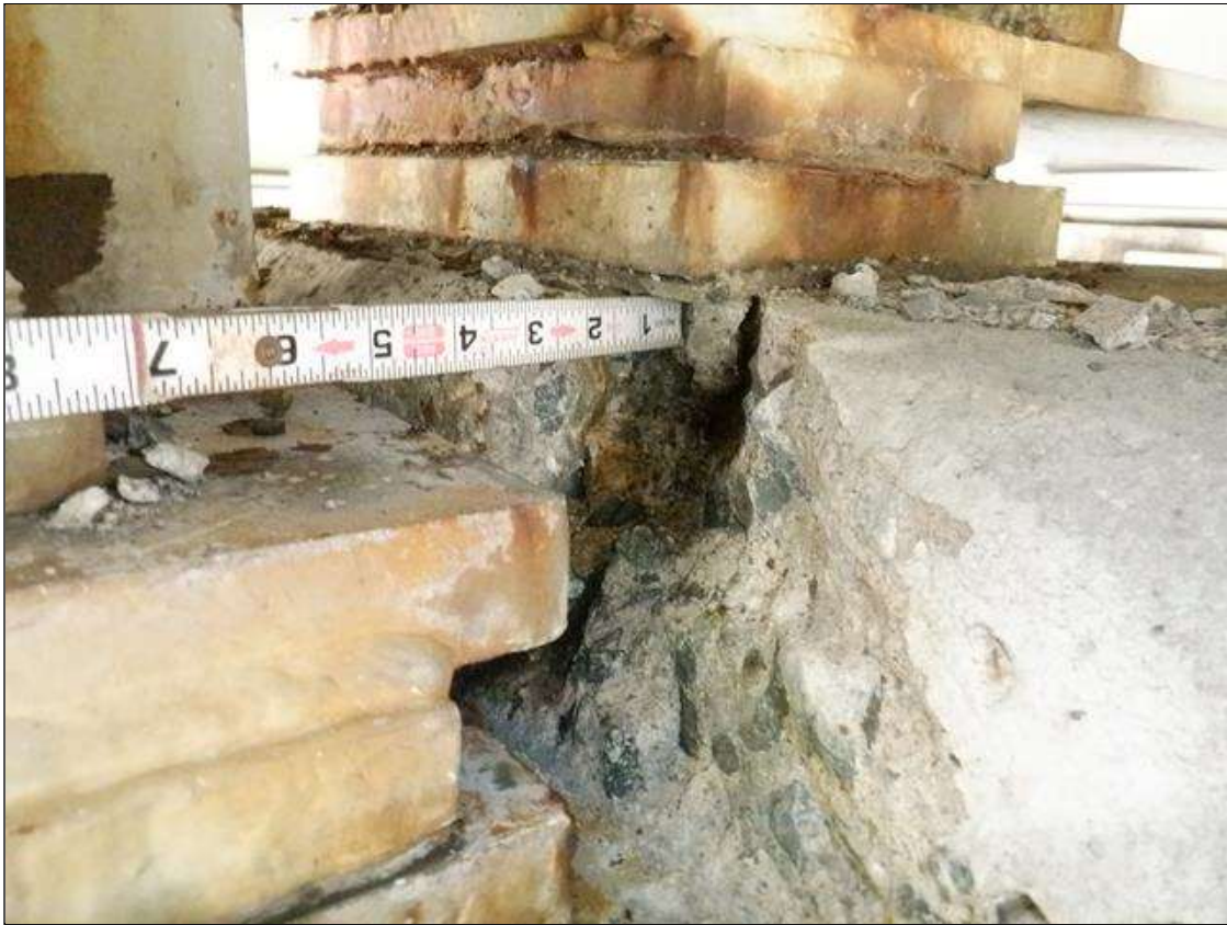
Bent 3 Cap 1: PAR: 6 INCH X 4 INCH X 5 INCH SPALL ON PEDESTAL UNDER GIRDER 5 SPAN 4 WITH 1 INCH X 1 1/2 INCH UNDER BEARING, NO EXPOSED REINFORCEMENT
