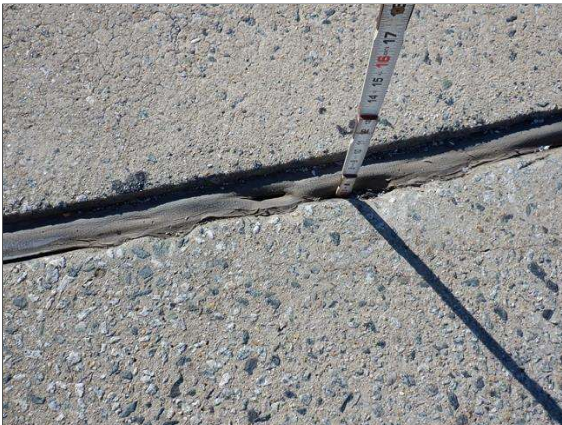
Span 2 Expansion Joint: WESTBOUND LANES, SEPARATION OF JOINT MATERIAL OVER BENT 1, UP TO FULL DEPTH OF FILLER MATERIAL
