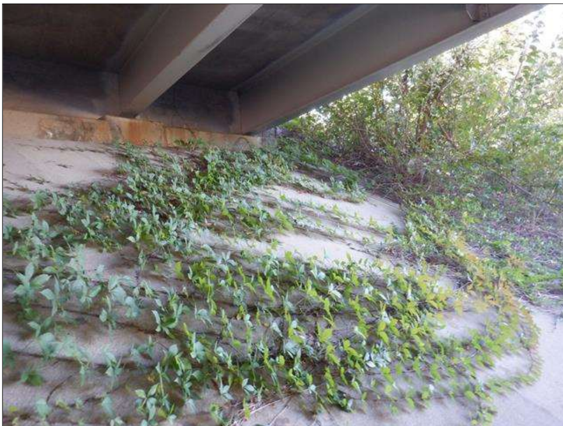
END BENT 2 SLOPE PROTECTION AT SOUTHEAST CORNER, 50 SQUARE FEET OF VEGETATION GROWTH
