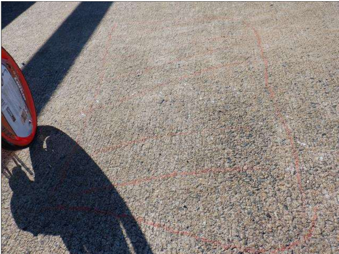
Span 2 Deck: 3 FEET WIDE DELAMINATION ALONG LEFT SHOULDER FOR ENTIRE SPAN LENGTH
