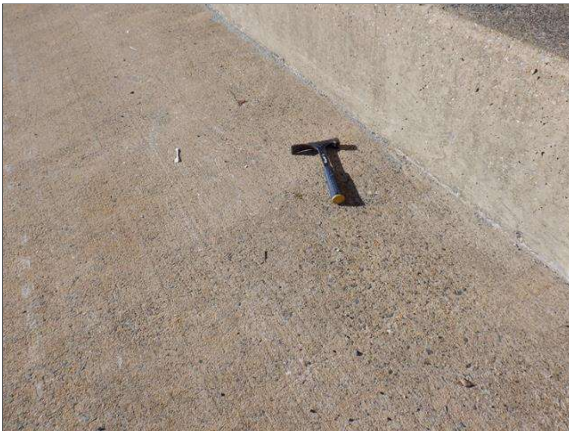
Span 2 Deck: MIDSPAN, ALONG RIGHT SHOULDER, 12 SQUARE FEET OF DELAMINATION
