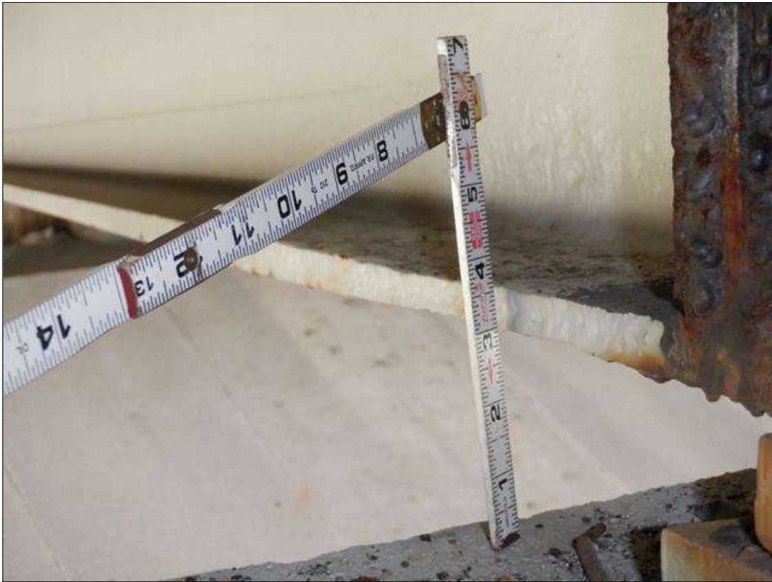
Span 4 Beam 3: CORROSION ARRESTED WITH PAINT, 3/16 INCH SECTION LOSS (9/16 INCH REMAINING) ON BOTH BOTTOM FLANGES FOR OUTER 2 INCH FOR 3 FEET STARTING 1.5 FEET FROM BENT 3 WITH 1/8 INCH SECTION LOSS (7/16 INCH REMAINING) ON LOWER 4 INCH OF WEB IN SAME AREA
