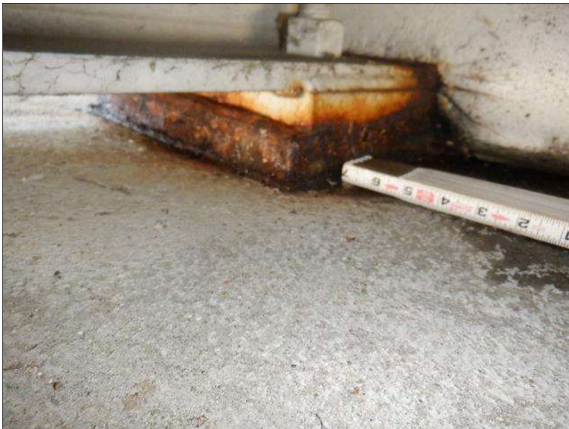
Span 4 Beam 1 - Far Bearing: CORROSION WITH PACK RUST, NO SECTION LOSS
