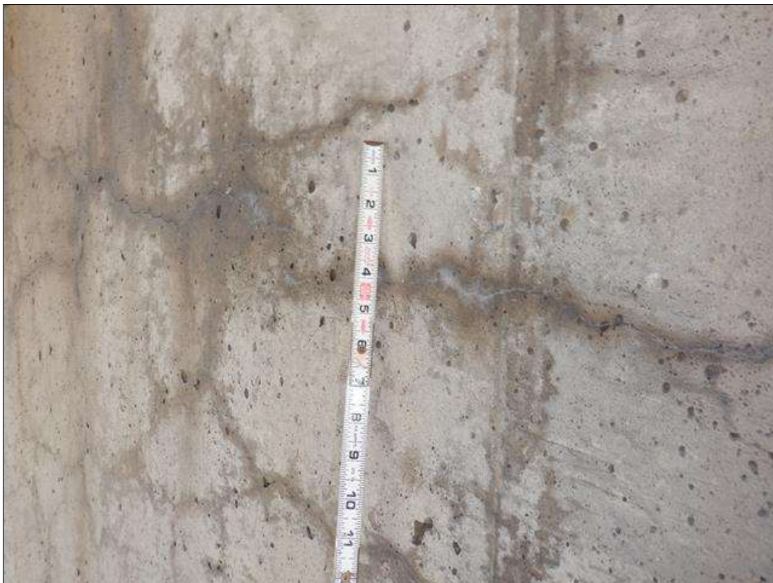
Bent 3 Cap 1: MAP CRACKING UP TO 1/16 INCH WIDE THROUGHOUT
