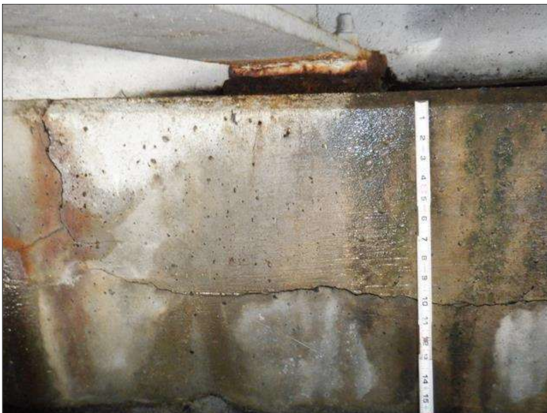
End Bent 2 Cap 1: BEAM 2 BEARING SEAT IS DELAMINATED FOR 1 FOOT LONG
