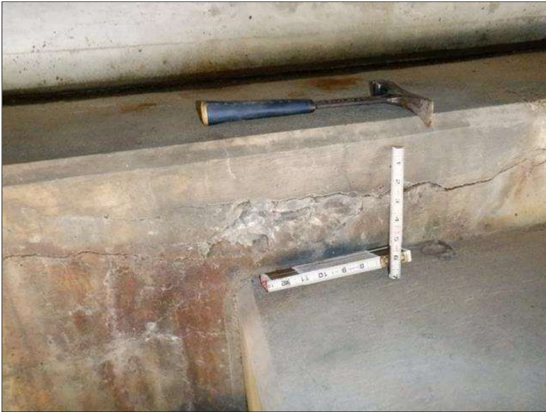
End Bent 2 Cap 1: 6 FEET LONG X 8 INCH HIGH DELAMINATION WITH RUST STAINING IN FACE OF CAP BELOW BAY 1 AND BAY 3 WITH 12 INCH X 3 INCH X 1/2 INCH DEEP SPALL BELOW BAY 3, NO EXPOSED REINFORCEMENT
