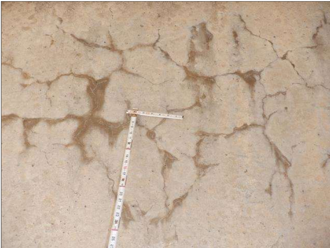
Bent 1 Cap 1: SCATTERED HAIRLINE MAP CRACKING THROUGHOUT FULL LENGTH OF CAP, UP TO FULL HEIGHT
