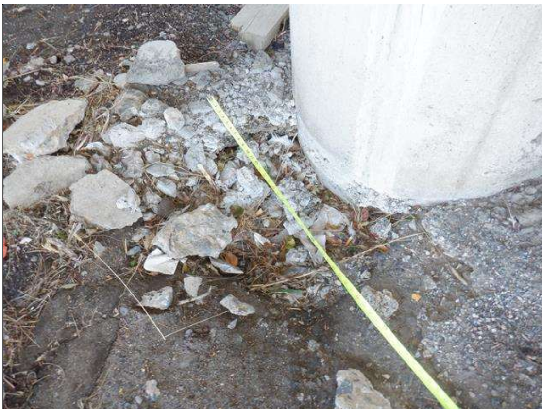
Bent 2 Pile 3: 20 INCH X 24 INCH X 10 INCH DEEP HOLE AT BASE OF PILE 3 ON WEST FACE
