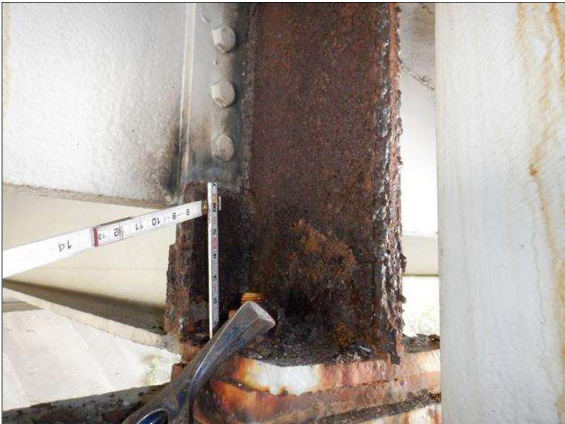
Span 4 Beam 5: WELDED STEEL PLATE REPAIR AT END OF BEAM BEHIND BEARING STIFFENER AT BENT 3, 6 INCH LONG X FULL HEIGHT
