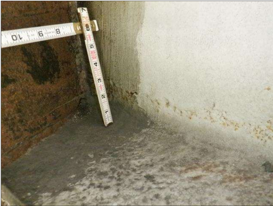
Span 3 Beam 5: CORROSION ARRESTED WITH PAINT, 1/2 INCH SECTION LOSS (3/4 INCH REMAINING) ON BOTH BOTTOM FLANGES FOR OUTER 2 INCH FOR 1 FOOT STARTING AT BENT 3
