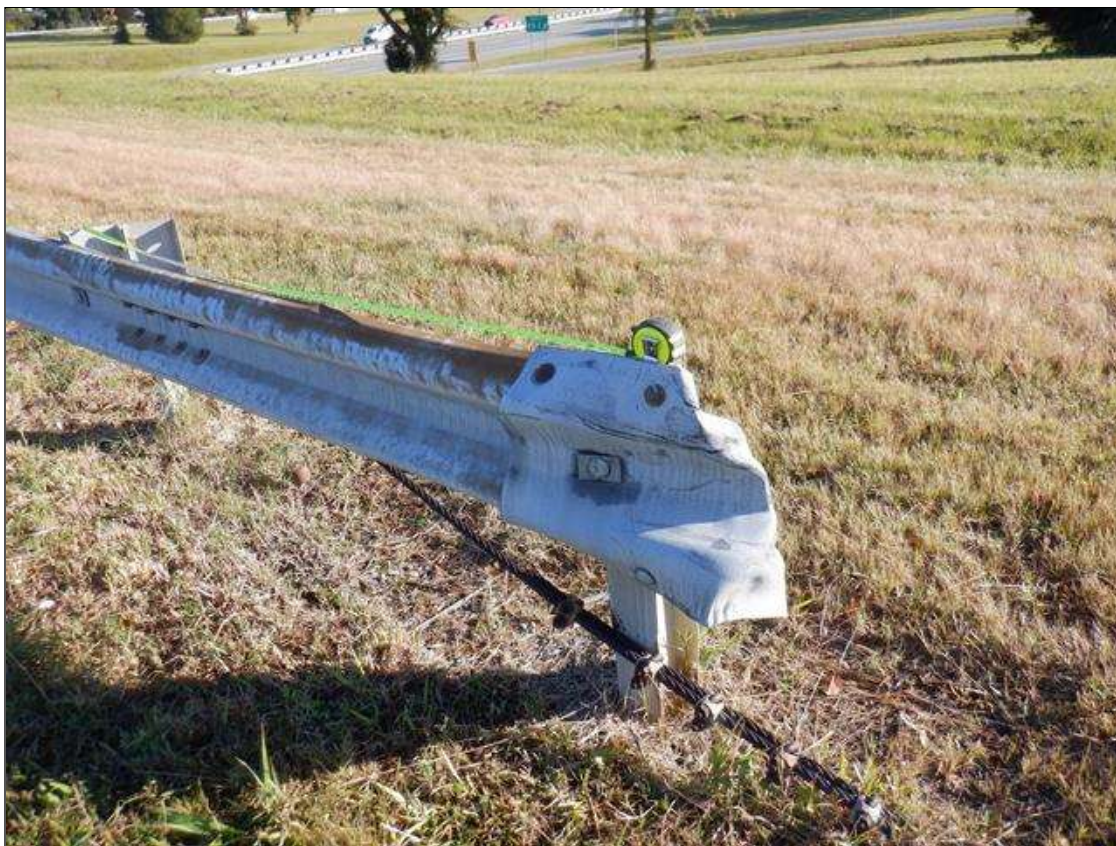
NORTHEAST GUARDRAIL TERMINAL, 1 FOOT OF IMPACT DAMAGE
