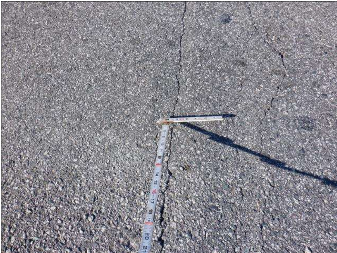
Span 3 Wearing Surface: SCATTERED TRANSVERSE CRACKING UP TO 1/16 INCH WIDE FOR 50 PERCENT OF PAVED JOINT LENGTH AT BENT 2
