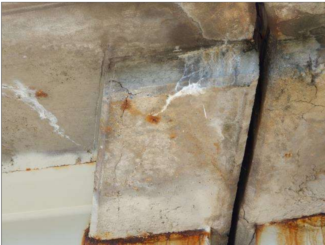
Span 2 Beam 1: AT BENT 1 LEFT OVERHANG DIAPHRAGM, DELAMINATION, 12 INCH X 6 INCH WITH EFFLORESCENCE
