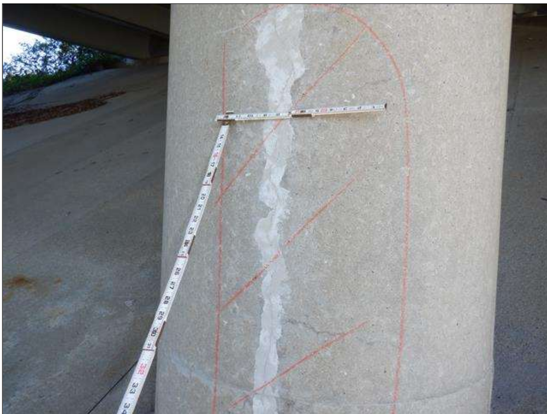
Bent 1 Pile 2: STARTING AT BOTTOM OF PILE ON EAST FACE, DELAMINATION 4 FOOT HIGH X 1 FOOT WIDE
