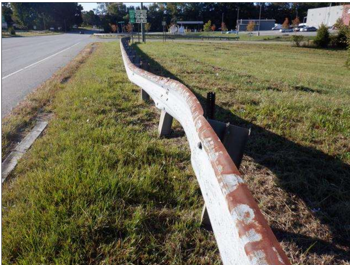
SOUTHEAST GUARDRAIL, STARTING 27 FEET FROM END BENT 2, 15 FEET OF IMPACT DAMAGE WITH UP TO 1 FOOT OF HORIZONTAL DISPLACEMENT
