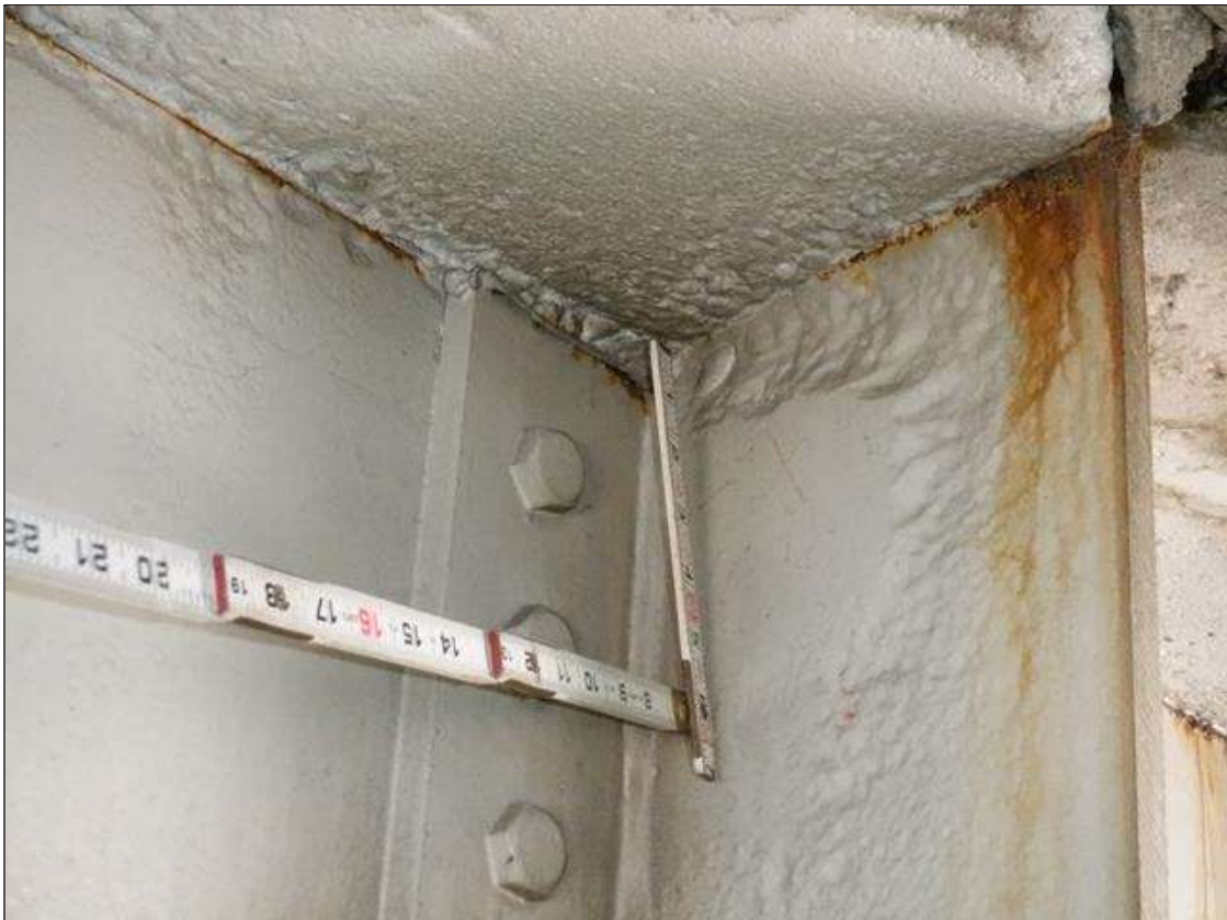
Span 4 Beam 6: CORROSION HAS BEEN ARRESTED WITH PAINT, 3/16 INCH SECTION LOSS (9/16 INCH REMAINING) ON TOP 6 INCH OF WEB FOR 10 INCH LONG AT BENT 3
