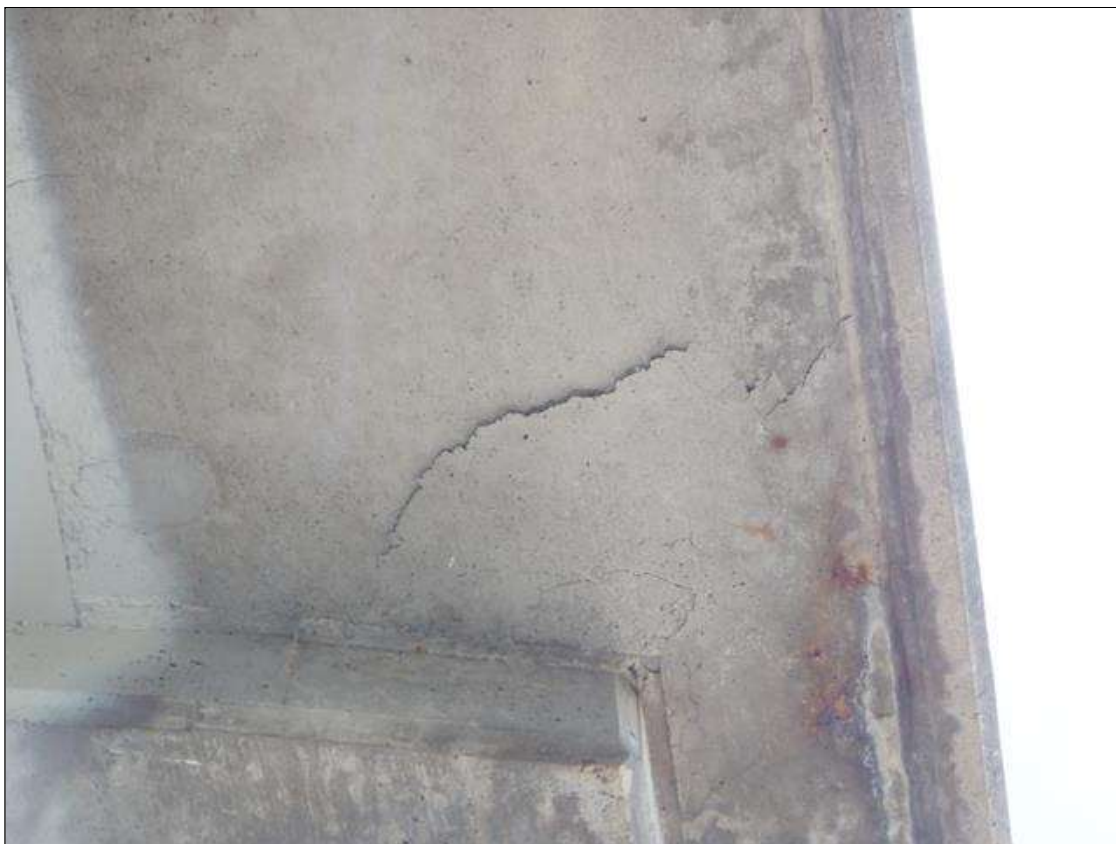
Span 4 Deck: BENT 3 LEFT OVERHANG SOFFIT, 8 INCH DIAMETER DELAMINATION
