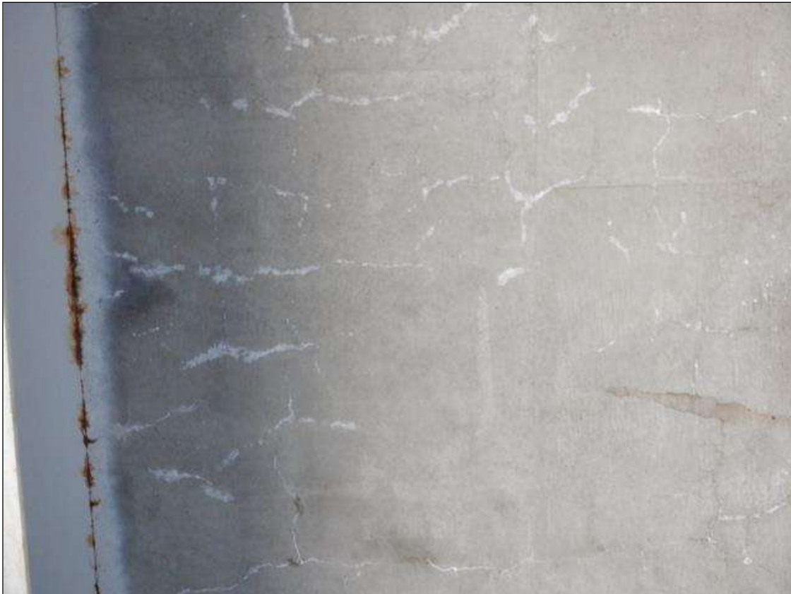
Span 2 Deck: HAIRLINE MAP CRACKING WITH EFFLORESCENCE SCATTERED THROUGHOUT UNDERSIDE
