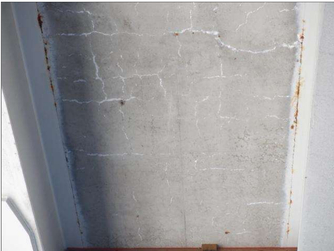
Span 3 Deck: THROUGHOUT UNDERSIDE IN ALL BAYS, HAIRLINE CRACKS WITH EFFLORESCENCE
