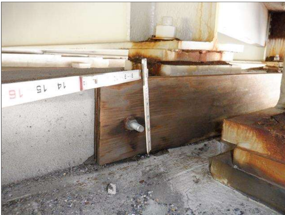
Bent 1 Cap 1: PATCHED PREVIOUS PRIORITY MAINTENANCE UNDER GIRDER 5 SPAN 1
