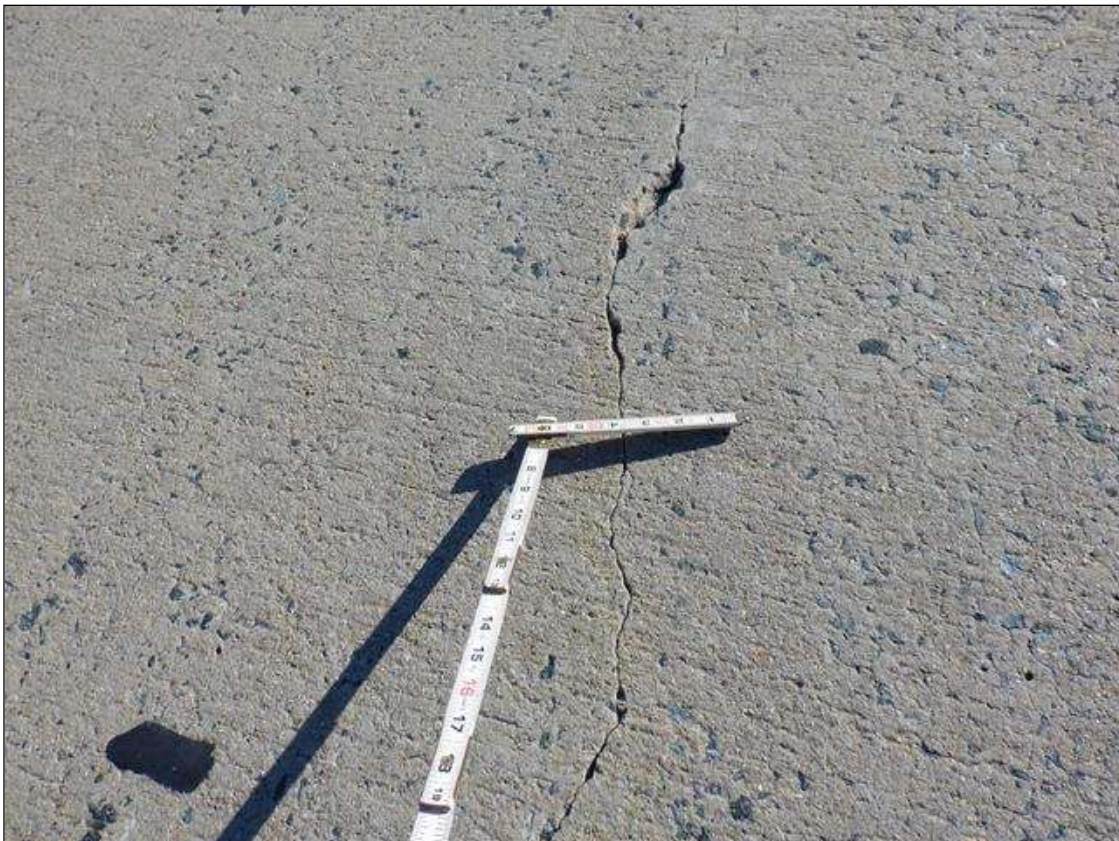
Span 4 Deck: 8 FEET TRANSVERSE CRACK UP TO 1/16 INCH WIDE IN FAR RIGHT EASTBOUND TRAVEL LANE NEAR END BENT 2
