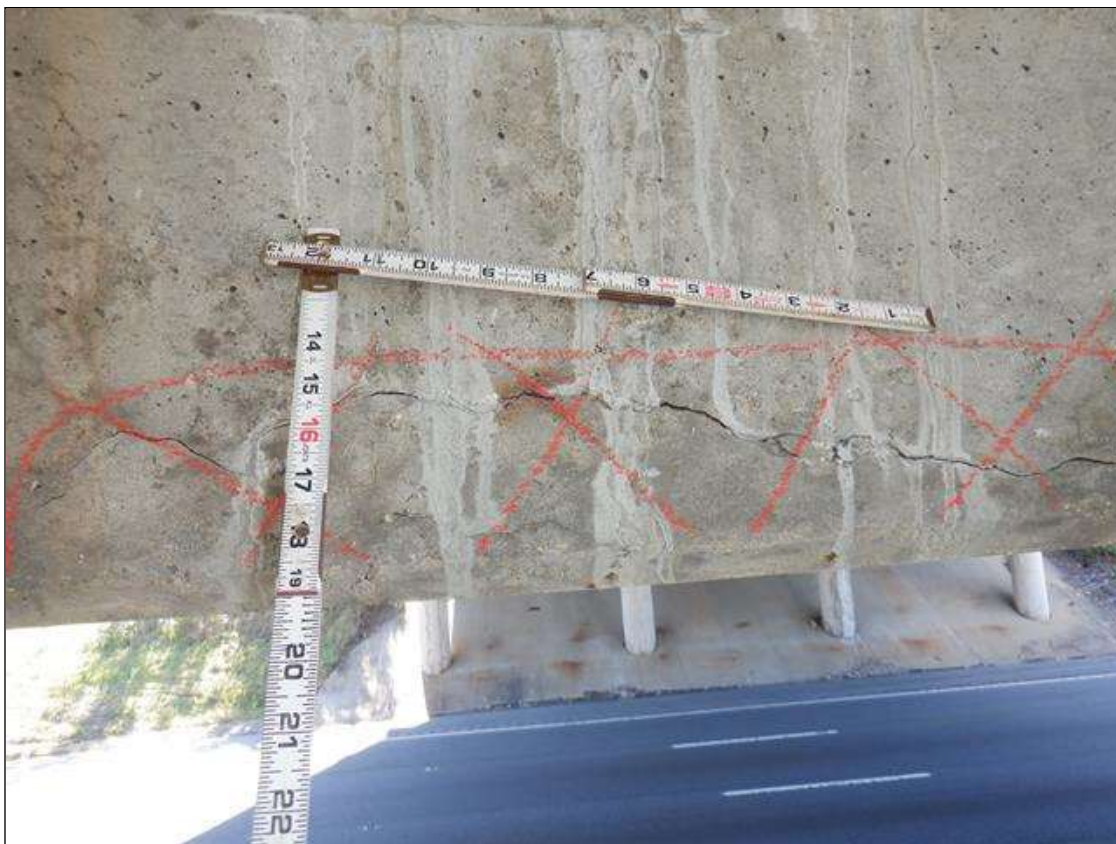
Bent 2 Cap 1: WEST FACE BELOW GIRDER 5 AT BOTTOM OF CAP, DELAMINATION 2 FOOT LONG X 6 INCH HIGH
