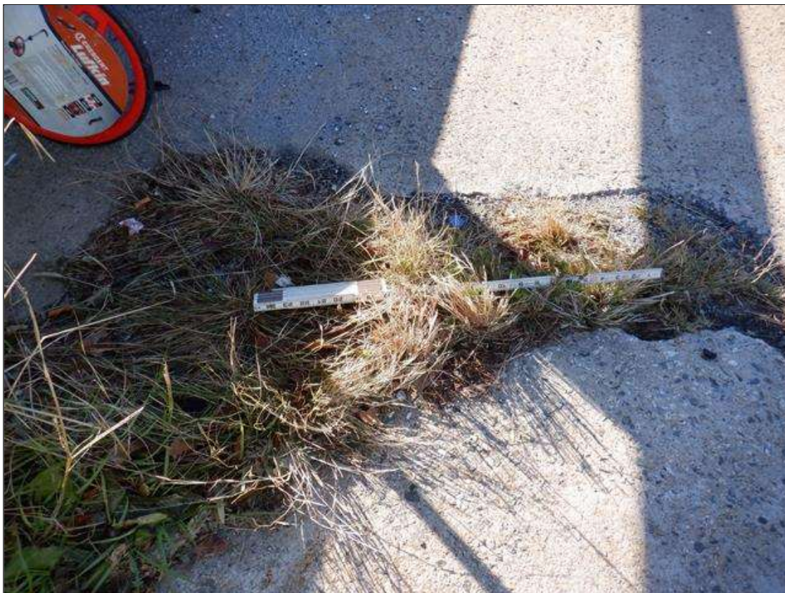
Span 3 Expansion Joint: LEFT SHOULDER, JOINT IS COMPLETELY FILLED WITH VEGETATION GROWTH
