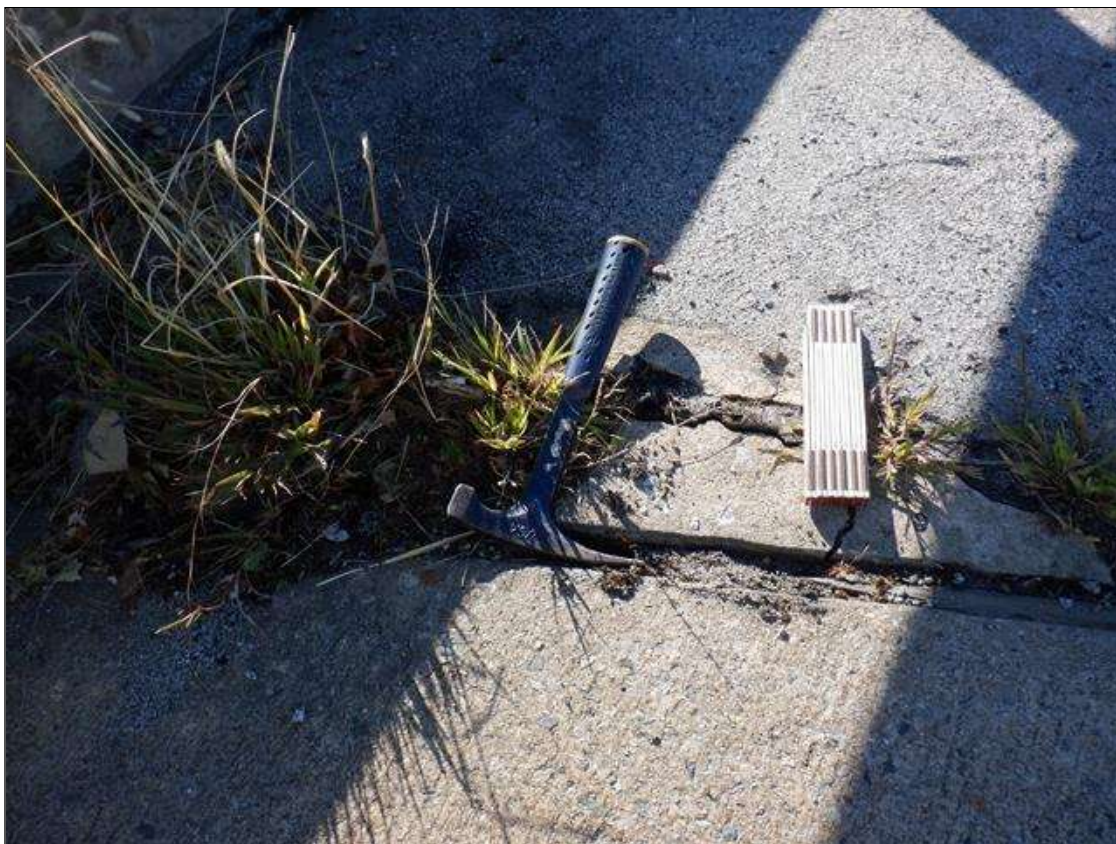
Span 2 Deck: 5 INCH X 9 INCH X 5 INCH DEEP SPALL ON LEFT SHOULDER AT BENT 1 JOINT, REBAR COVERED BY PACKED DEBRIS
