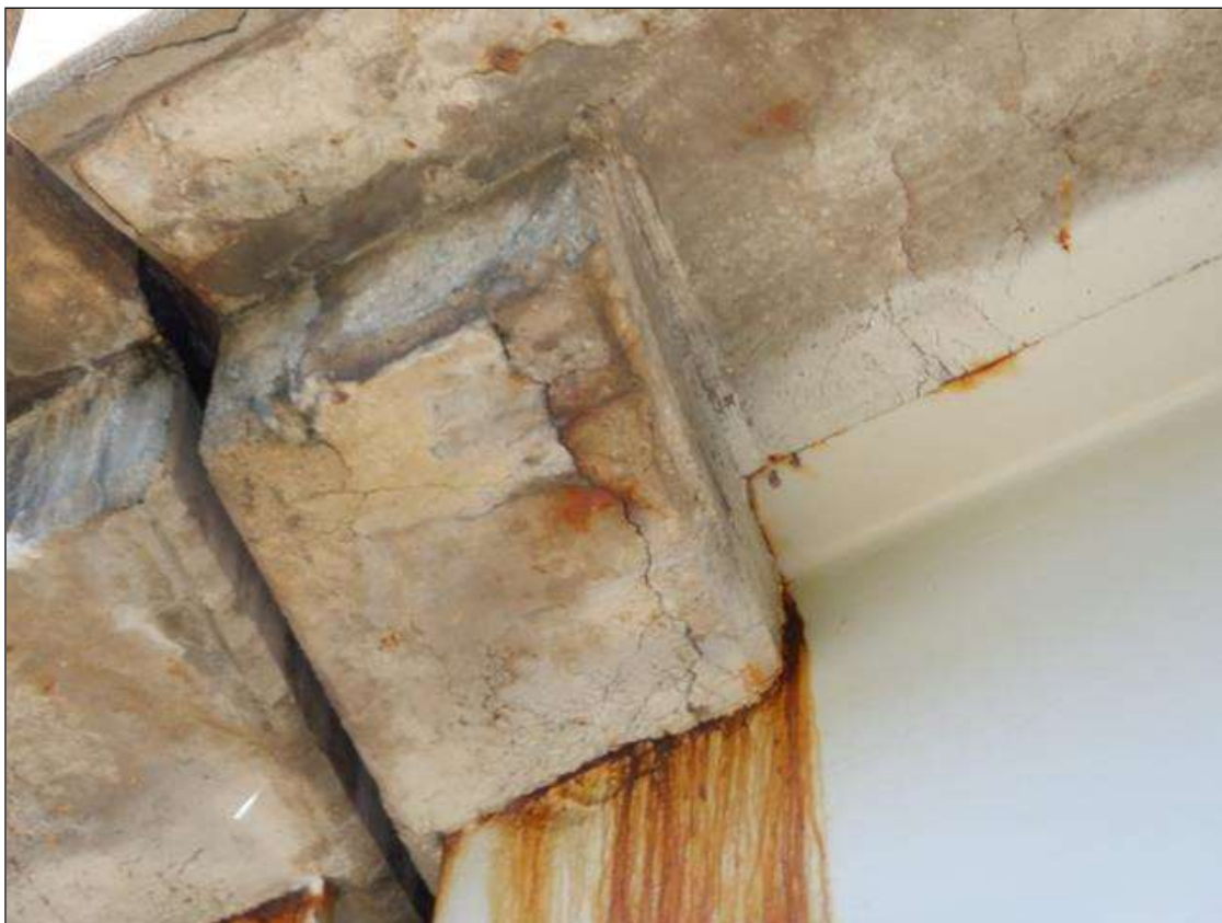
Span 1 Beam 1: AT BENT 1 LEFT OVERHANG DIAPHRAGM, DELAMINATION, 12 INCH X 6 INCH WITH RUST STAINS
