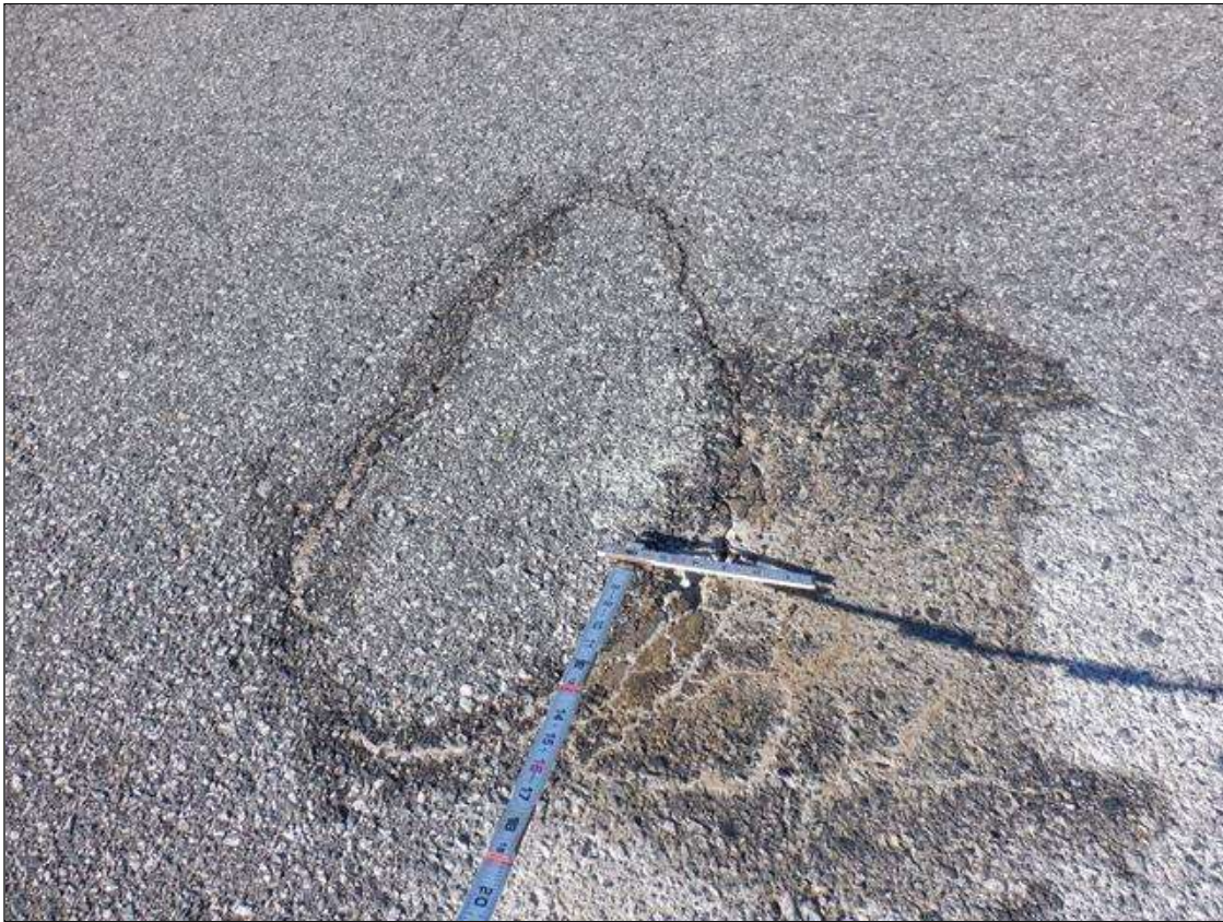
Span 3 Wearing Surface: WESTBOUND LANE, 10 FEET FROM BENT 2, 2 POTHOLES UP TO 2 FOOT DIAMETER WITH ADJACENT CRACKS UP TO 1/16 INCH WIDE
