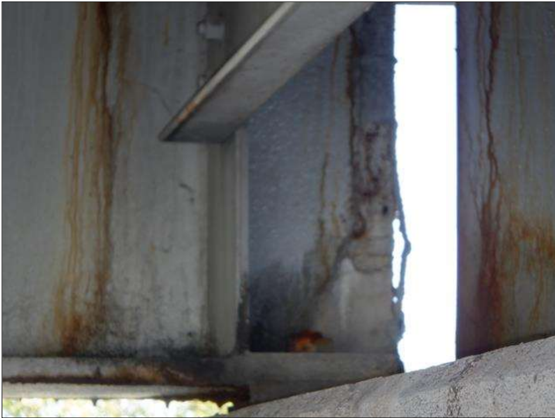
Span 3 Beam 1: CORROSION WITH 1/16 INCH SECTION LOSS FULL HEIGHT OF WEB AT END OF BEAM
