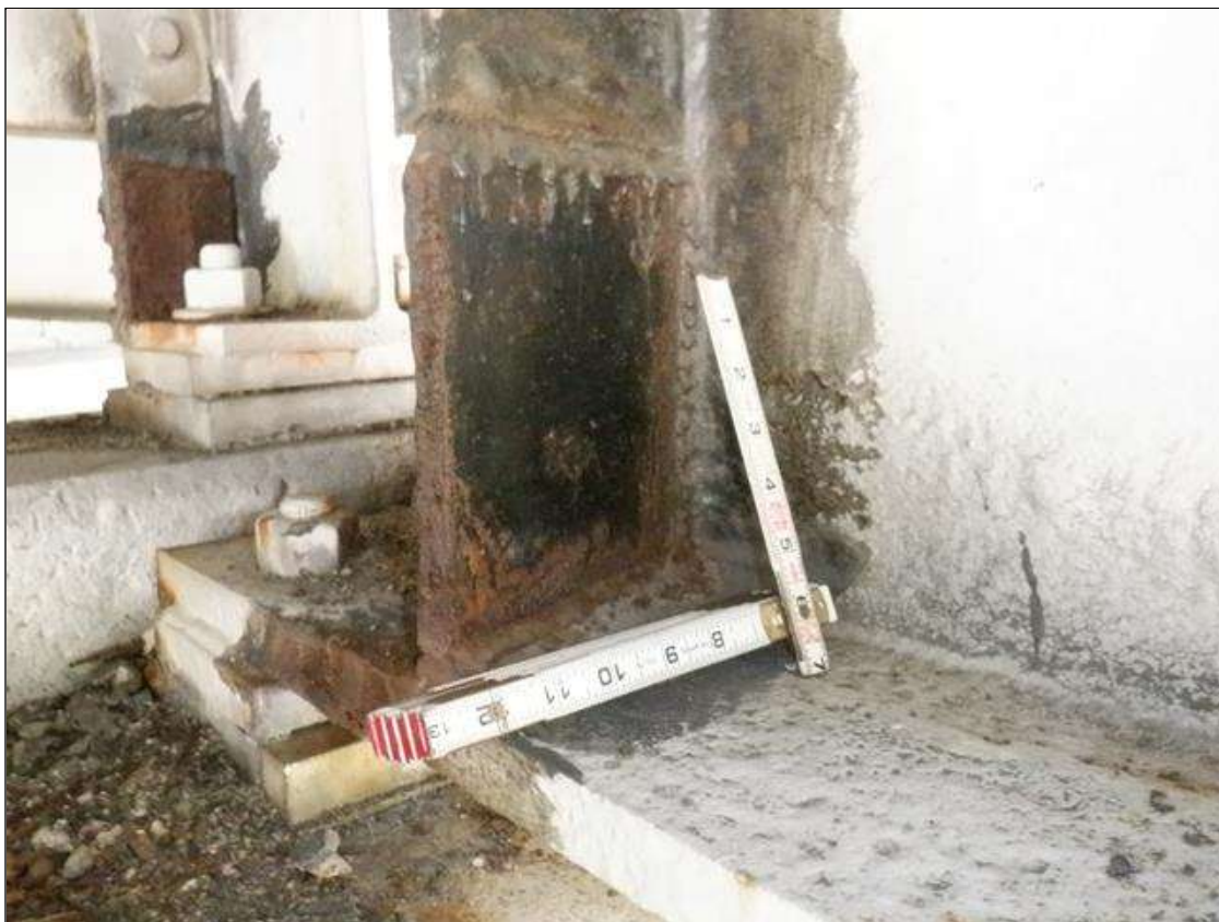
Span 3 Beam 6: WELDED PLATE REPAIR TO BOTH SIDES OF LEFT BEARING STIFFENER AT BENT 3, 5 INCH HIGH X 4 INCH WIDE X 3/8 INCH THICK WITH RUST SCALE
