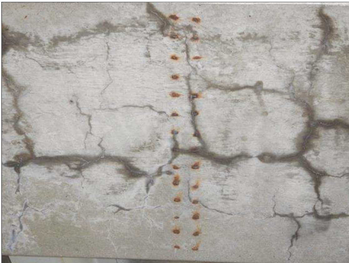
Bent 3 Cap 1: ALONG SOFFIT, 9 FEET OF EXPOSED REBAR CHAIRS
