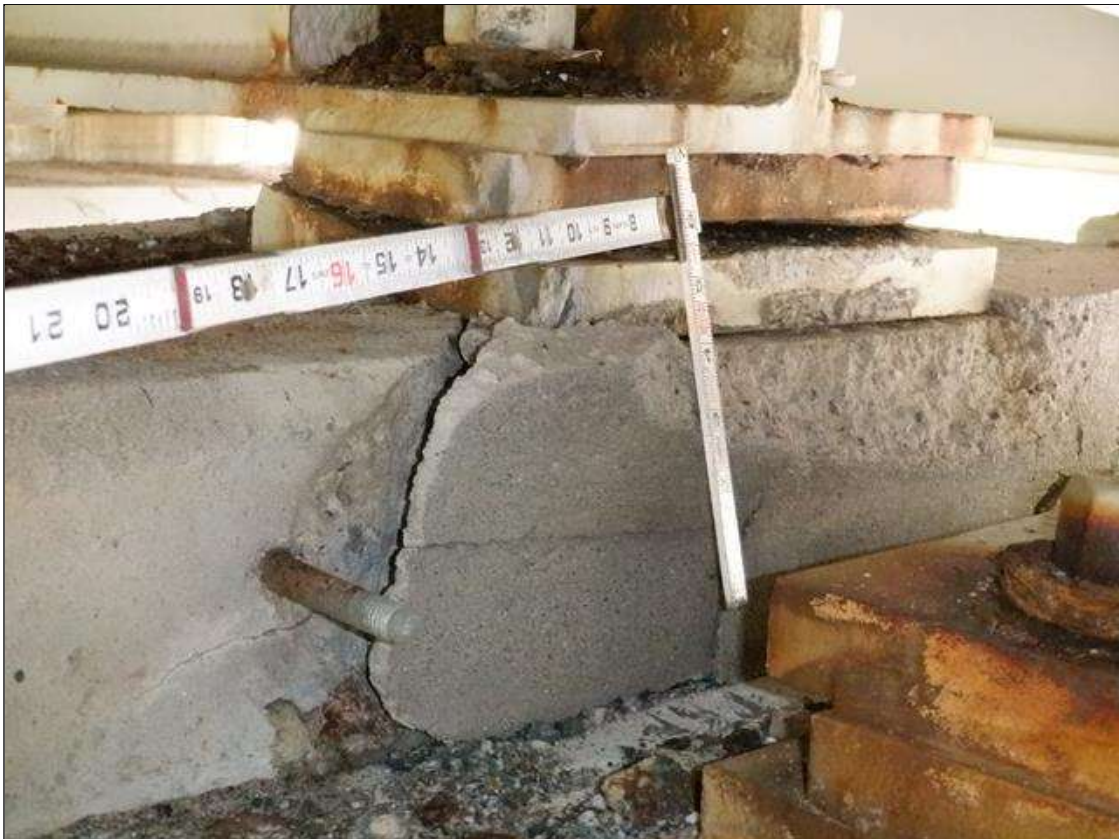
Bent 1 Cap 1: 14 INCH X 3 INCH X 1 INCH DEEP SPALL ON PEDESTAL UNDER GIRDER 4 SPAN 1 WITH NO LOSS OF BEARING AT EAST END OF BEAM, NO EXPOSED REINFORCEMENT
