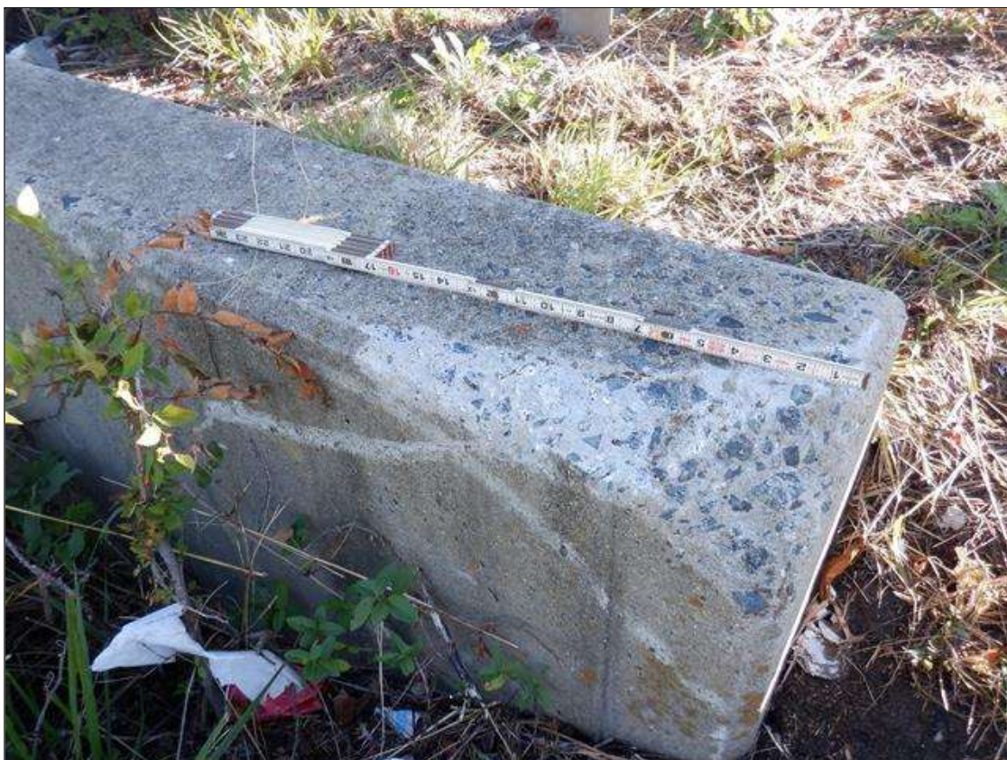
SOUTHEAST WINGWALL, ALONG TOP, 4 SPALLS UP TO 16 INCH LONG X 6 INCH WIDE X 1 INCH DEEP
