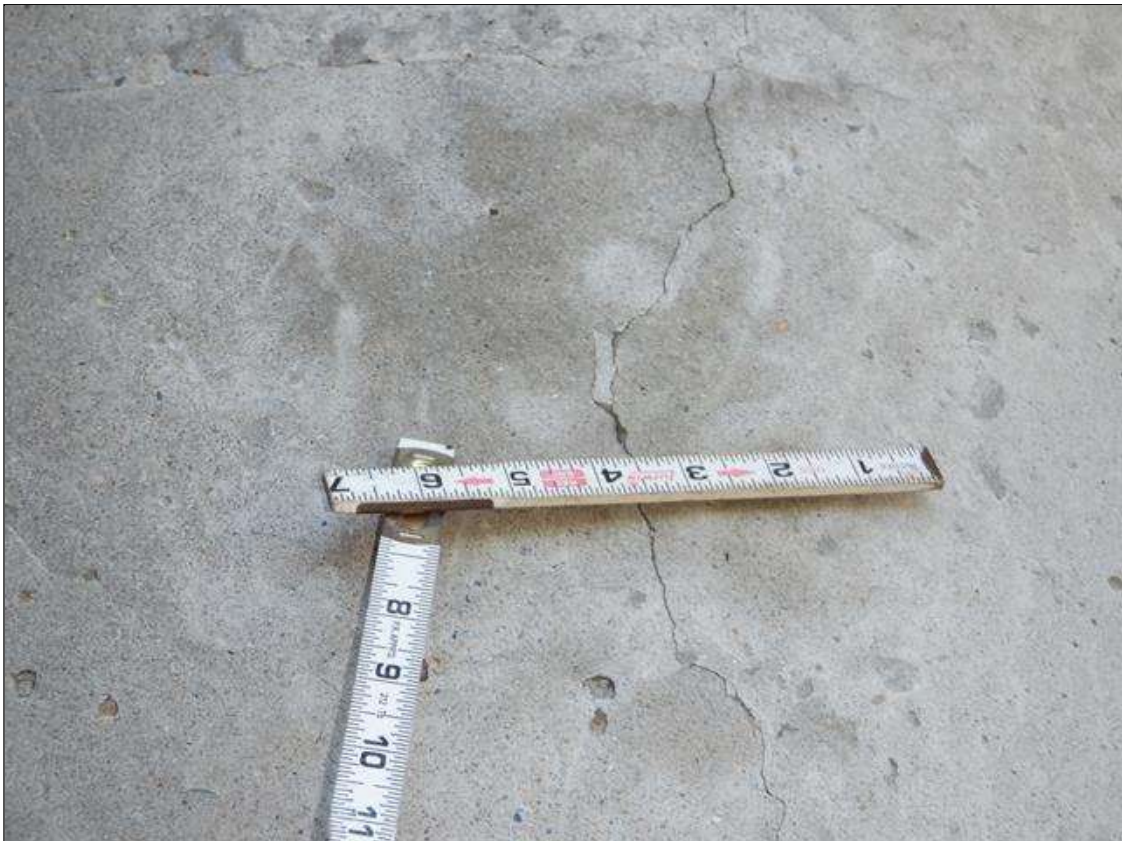
Bent 1 Pile 4: 8 FEET OF CRACKING UP TO 1/16 INCH WIDE
