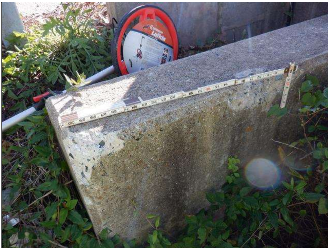
SOUTHWEST WINGWALL AT TOP CORNER, 2 SPALLS, UP TO 1 FOOT LONG X 5 INCH HIGH X 1 INCH DEEP
