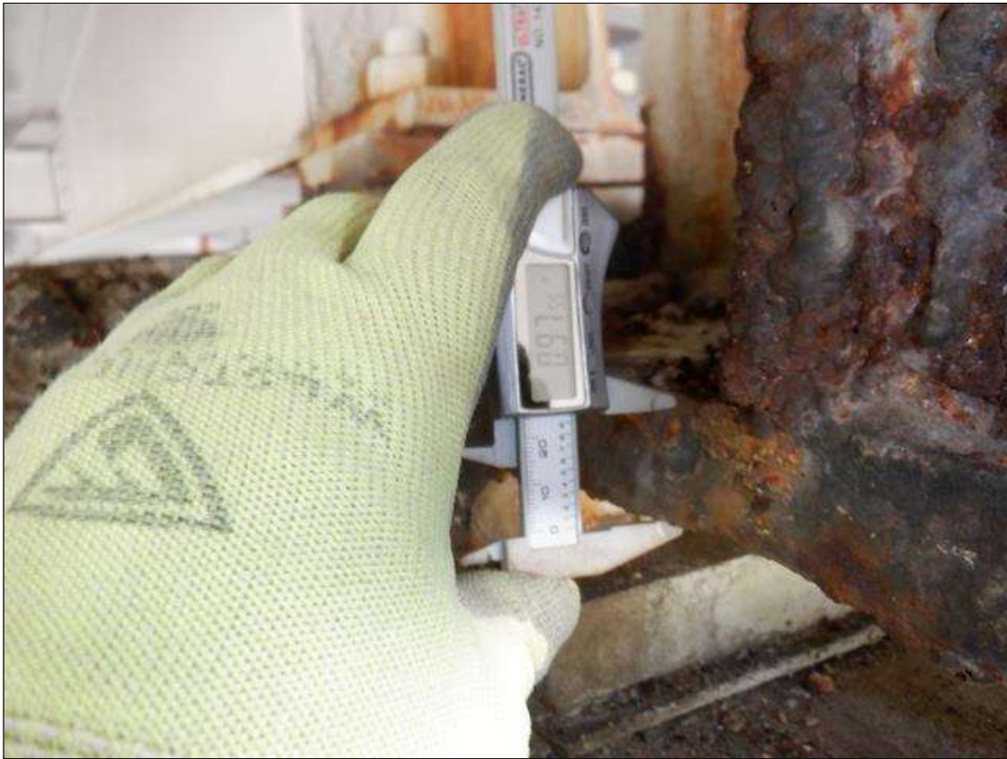
Span 3 Beam 4: PAR: CORROSION WITH 5/16 INCH SECTION LOSS (15/16 INCH REMAINING) ON LEFT BOTTOM FLANGE FOR OUTER 2 INCH FOR 9 INCH LONG STARTING 7 INCH FROM BENT 3
