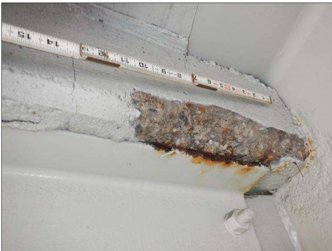
Span 2 Beam 5: BENT 1 BAY 5 DIAPHRAGM, SPALL, 10 INCH X 3 INCH X 1 INCH DEEP
