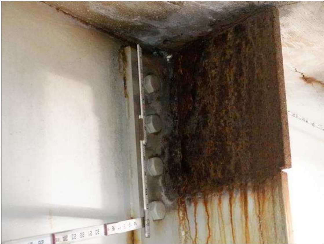
Span 1 Beam 4: AT BENT 1, TOP 9 INCHES OF WEB HAS A REPAIR PLATE, 9 INCH HIGH X 9 INCH LONG X 1/2 INCH THICK WITH RUST SCALE
