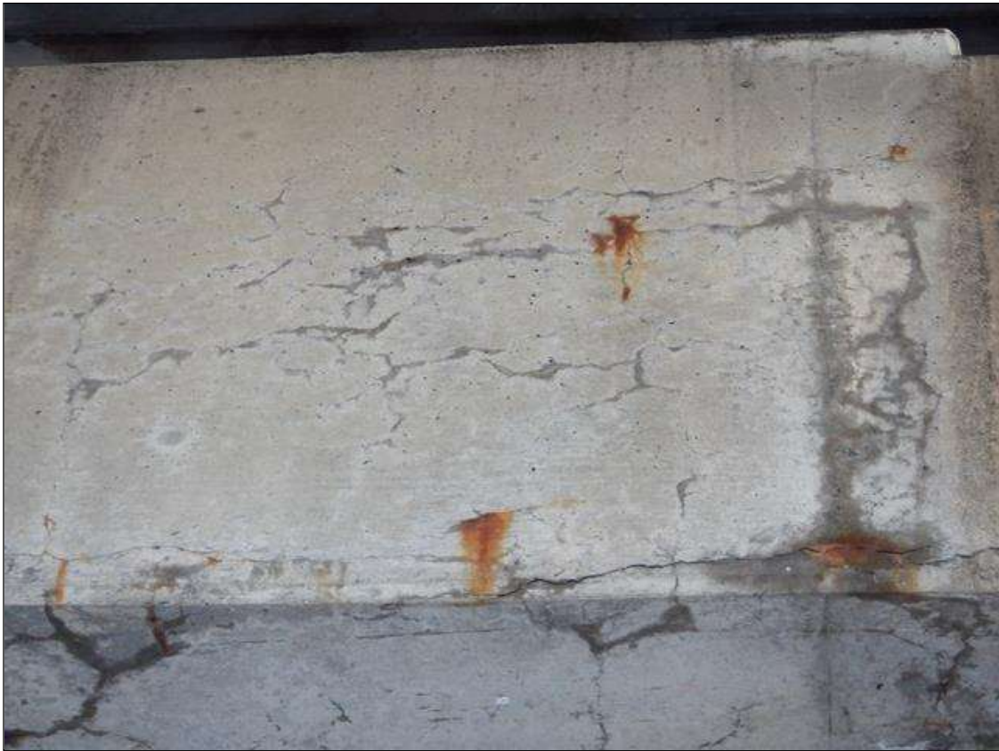
Bent 1 Cap 1: EAST FACE, BELOW GIRDER 7, DELAMINATED AREA UP TO 6 FOOT LONG X 2 FOOT HIGH WITH HAIRLINE CRACKS AND RUST STAINING
