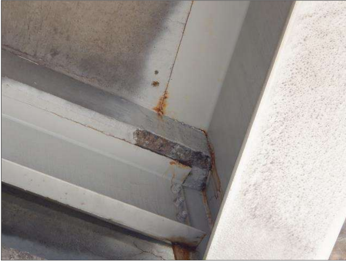
Span 2 Beam 1: AT BENT 1 BAY 1 DIAPHRAGM, SPALL, 1 FOOT LONG X 2 INCH HIGH X 1 INCH DEEP
