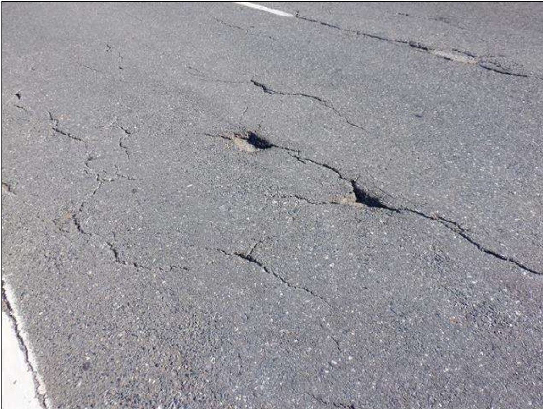
WEST APPROACH ASPHALT WEARING SURFACE HAS LONGITUDINAL CRACKS UP TO 1/4 INCH WIDE WITH POTHOLES UP TO 6 INCH DIAMETER X 1 INCH DEEP
