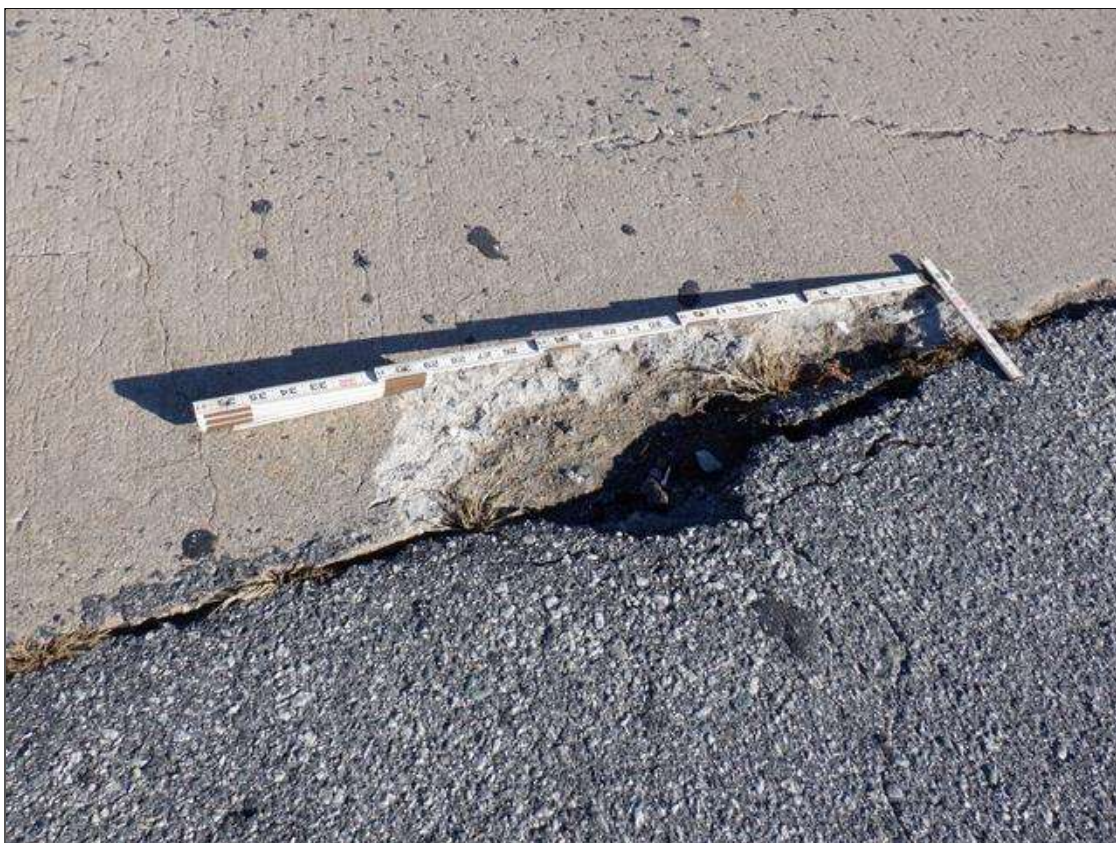
Span 4 Deck: EASTBOUND LANE AT END BENT 2, SPALL, 18 INCH WIDE X 8 INCH LONG X UP TO 1 INCH DEEP
