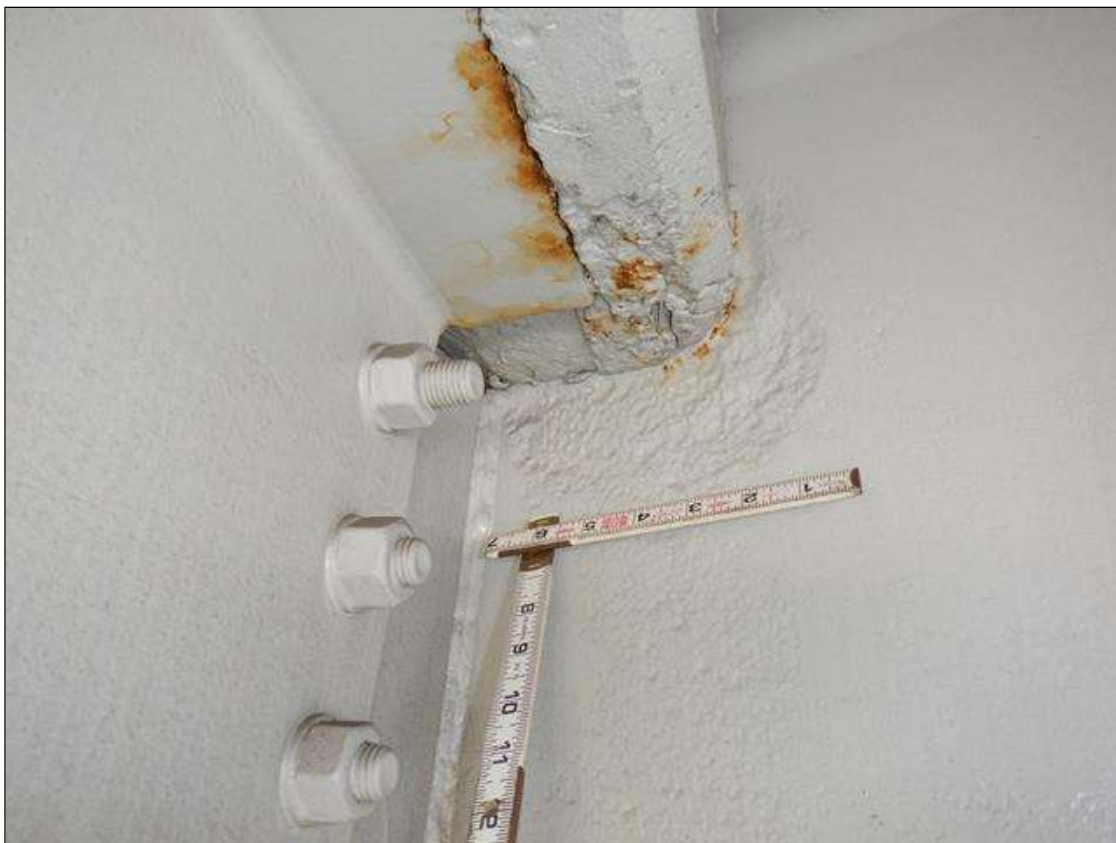
Span 2 Beam 5: 3/16 INCH SECTION LOSS (9/16 INCH REMAINING) ON LOWER 10 INCH AND TOP 3 INCH OF WEB FOR 10 INCH LONG AT BENT 1. CORROSION HAS BEEN ARRESTED
