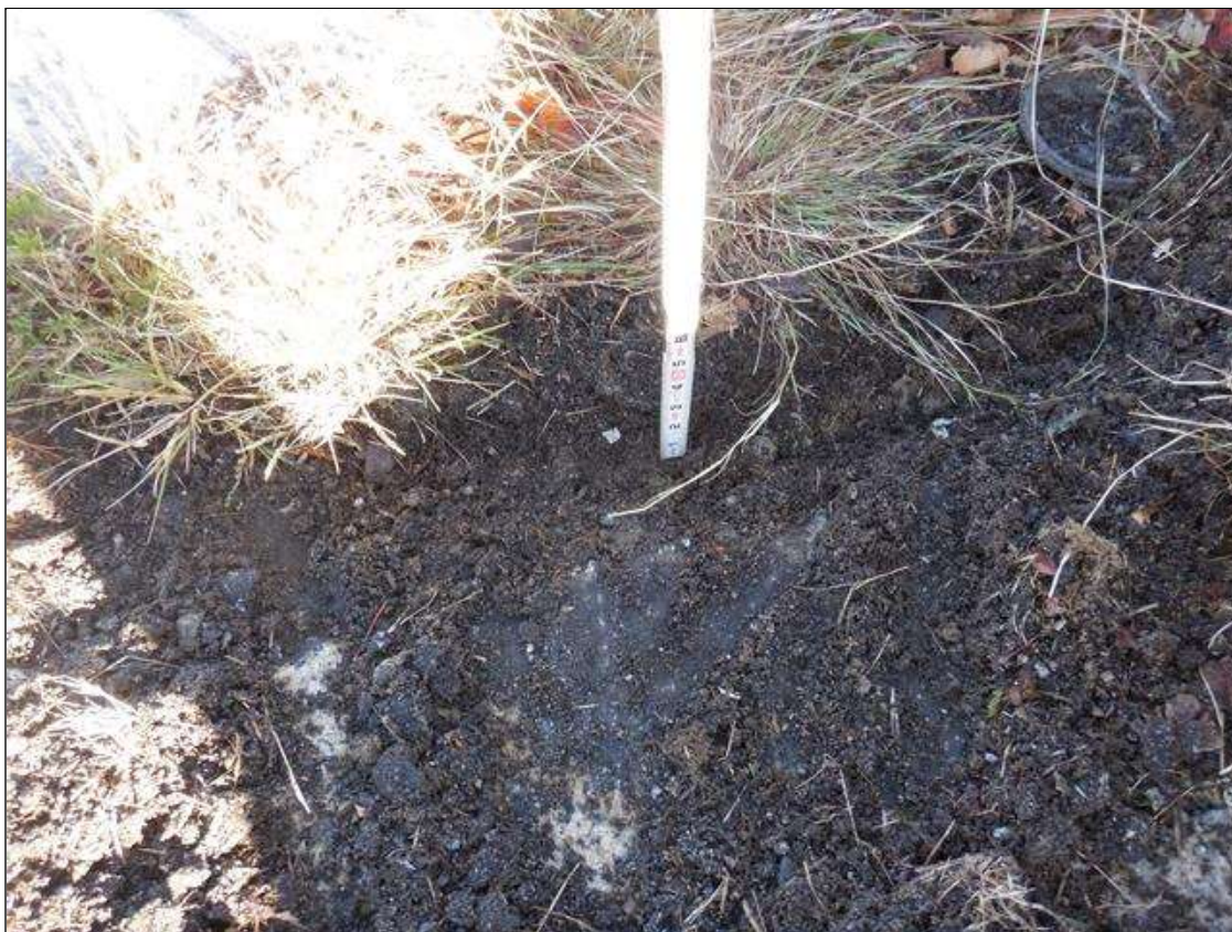
Span 3 Deck: UP TO 4 FEET X 1 FOOT X 5 INCH DEEP SPALL ON LEFT SHOULDER AT BENT 2 JOINT, REBAR COVERED BY PACKED DEBRIS
