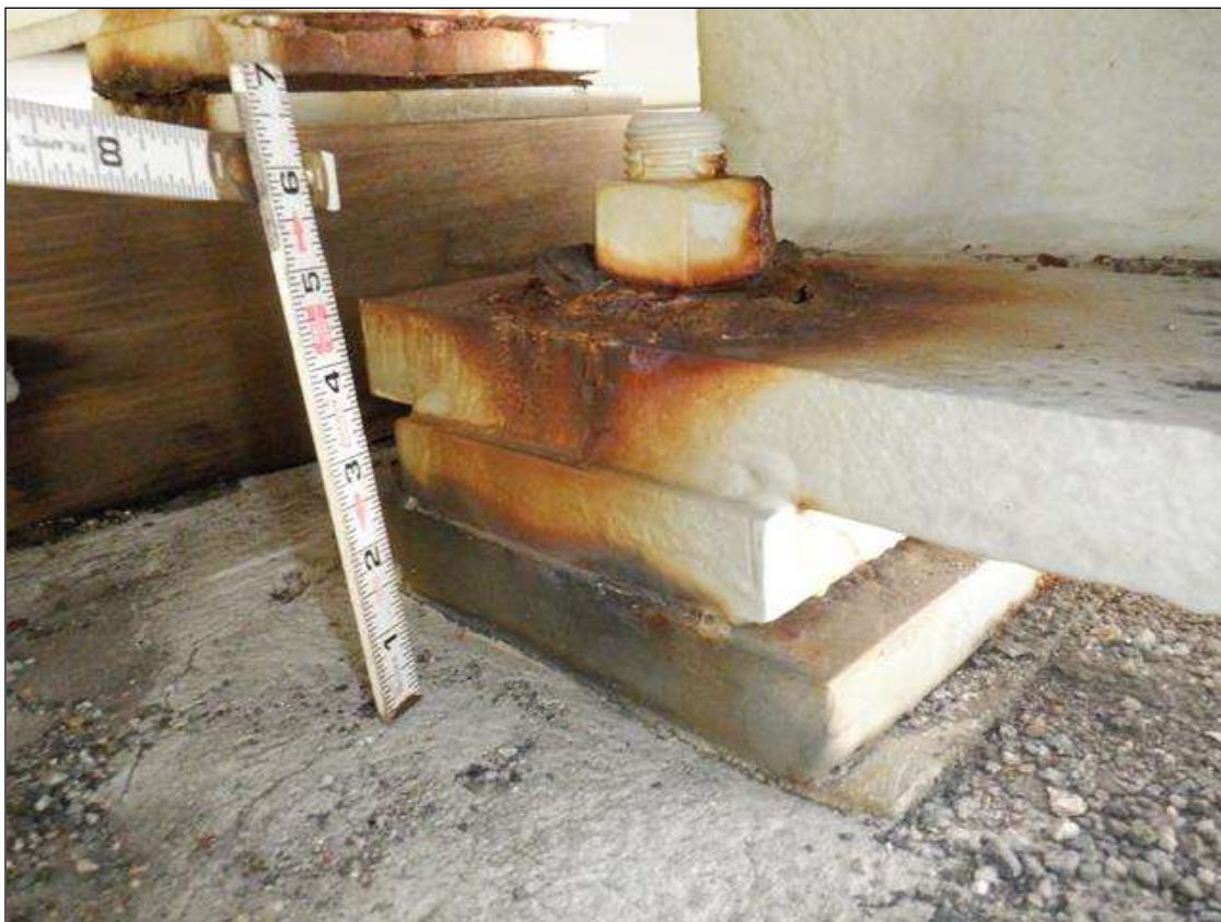
Span 2 Beam 5 - Near Bearing: FRECKLED RUST ON BEARING PLATES
