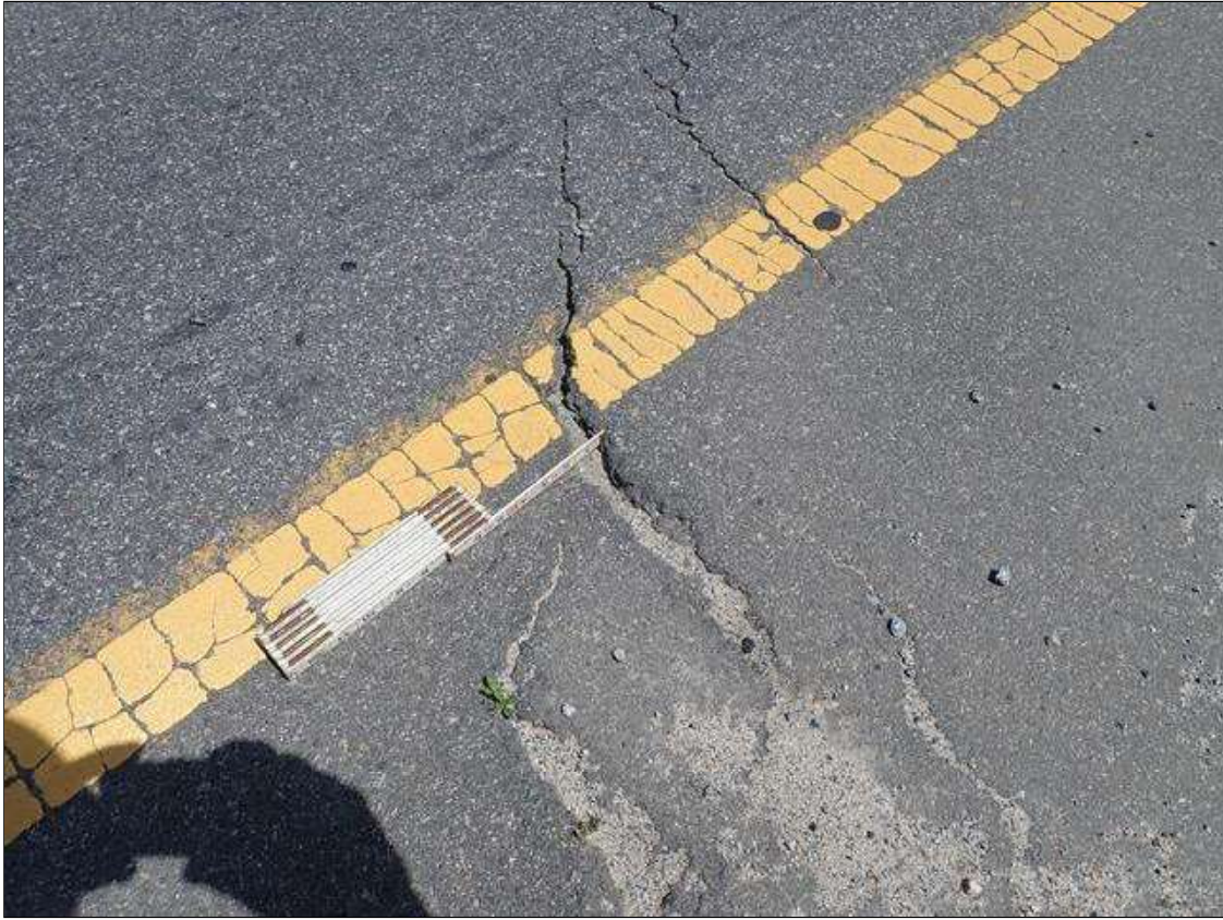
Span 1 Wearing Surface: AT THE SPAN ENDS, SCATTERED TRANSVERSE CRACKING UP TO 1" WIDE
