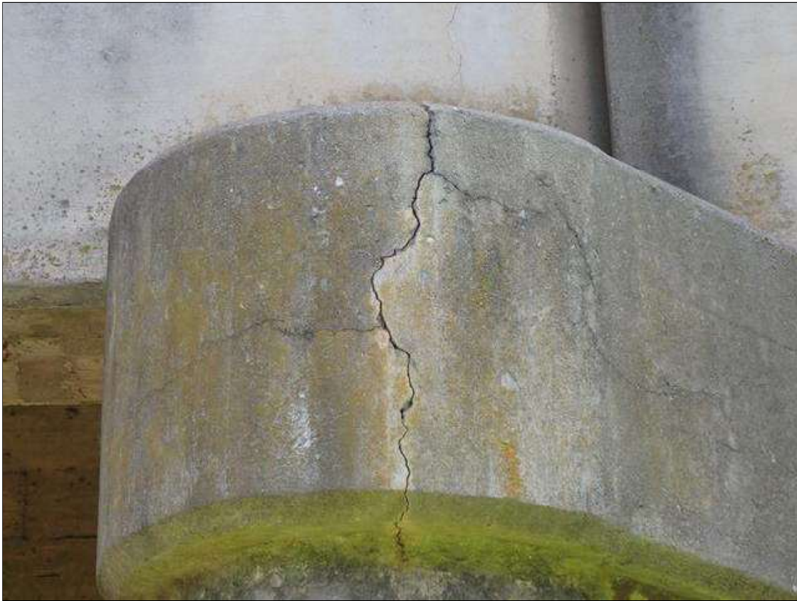
Bent 1 Cap 1: east face, map cracking (full height x full width x 1/8")
