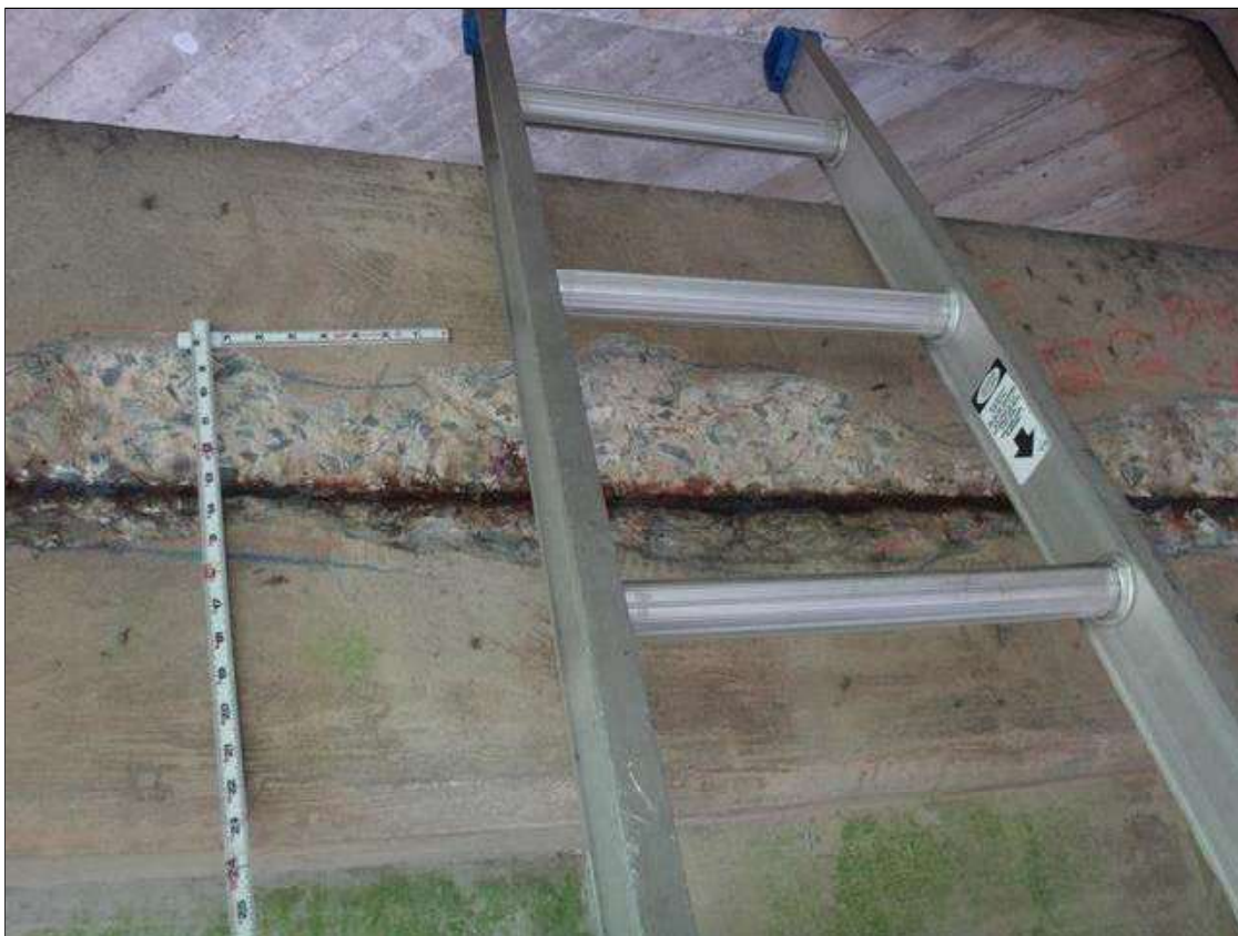
Bent 2 Cap 1: [PAR] north face at bay 2, spall (5' x 10" x 1.75") with exposed rusted rebar [section loss up to 1/8"]
