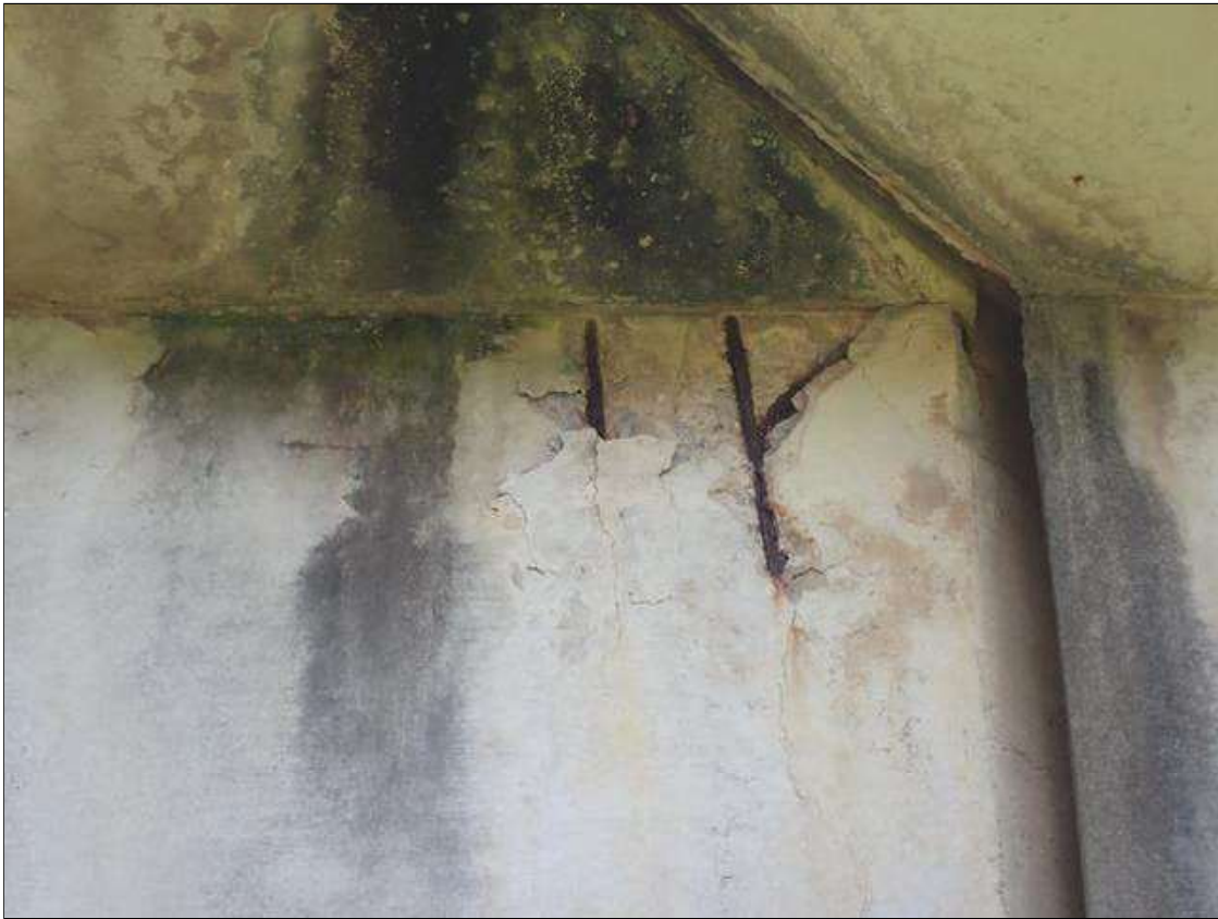
Span 2 Beam 1: GIRDER END AT BENT 1, LEFT SIDE AT THE TOP, SPALL WITH EXPOSED REBAR [APPROXIMATELY 18" DIAMETER X UP TO 3/4" DEEP], NO MEASURABLE SECTION LOSS. adjacent delamination [2' x up to 18" high]
