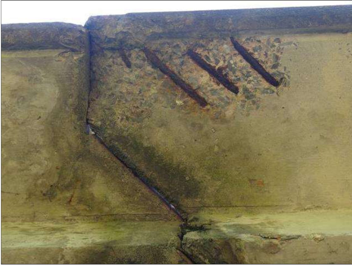
Span 2 Deck: underside east overhang at bent 1, spalls (up to 1' x 8" x 1") with exposed rusted rebar, NO MEASURABLE SECTION LOSS
