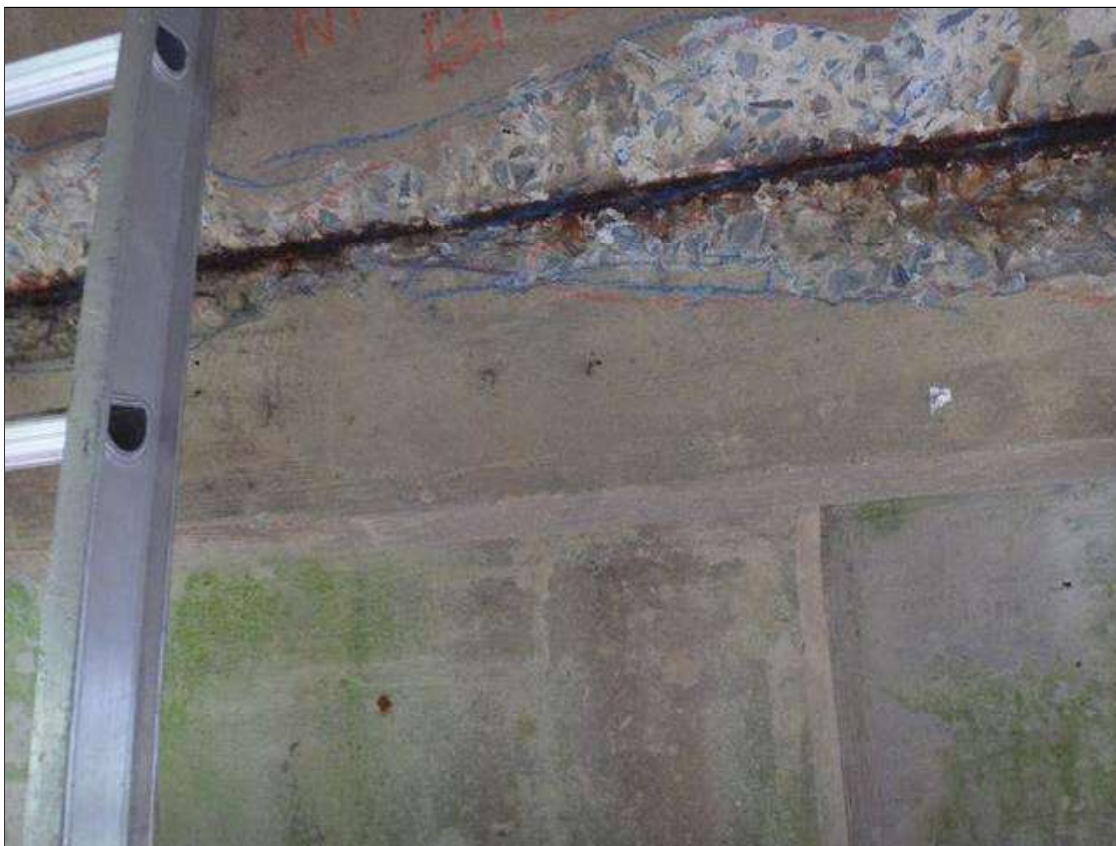
Bent 2 Cap 1: [PAR] north face at bay 2, spall (5' x 10" x 1.75") with exposed rusted rebar [section loss up to 1/8"]
