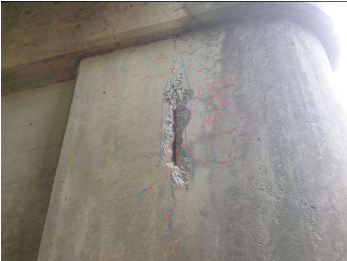
Bent 1 Pile 1: [PAR] North face, approximately 3' below cap, spall [32" x 4" x 1" deep] with exposed rusted reinforcing with no measurable section loss
