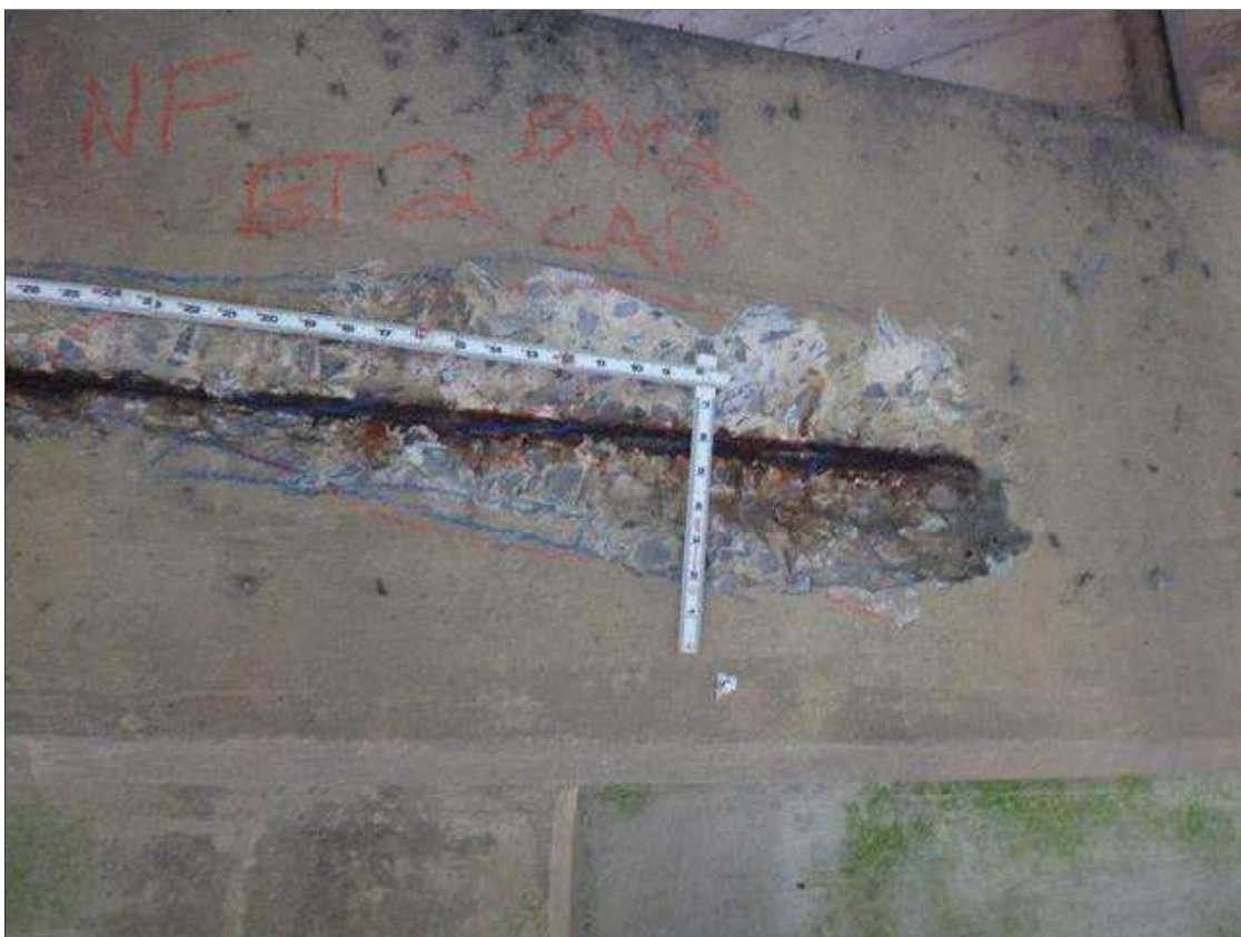
Bent 2 Cap 1: [PAR] north face at bay 2, spall (5' x 10" x 1.75") with exposed rusted rebar [section loss up to 1/8"]
