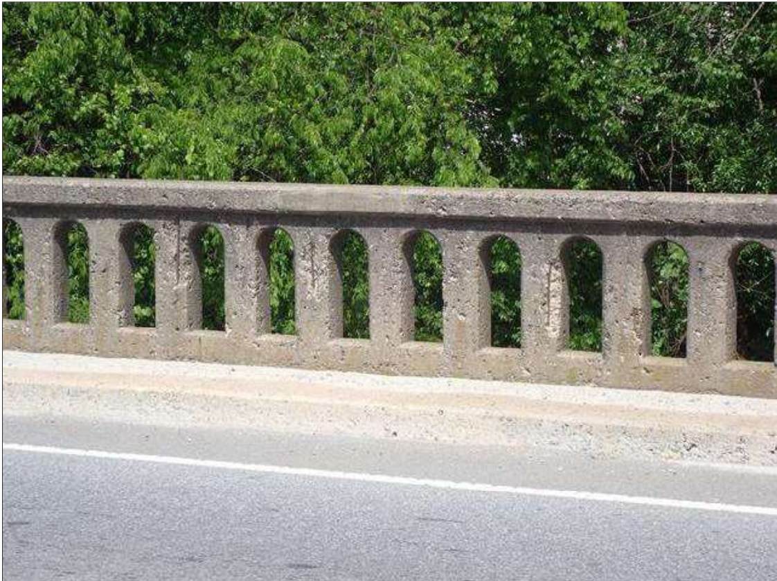
Span 1 Right Bridge Rail: near bent 1, (3) spalls (up to 15" x 5" x 1") with exposed rusted rebar, [loss up to 1/8"]
