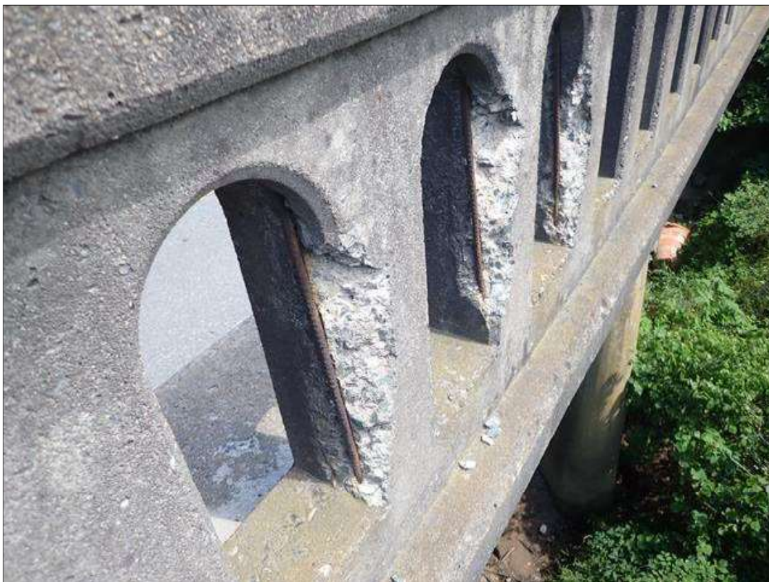
Span 2 Left Bridge Rail: exterior face at 13ft from bent 1, (3) spalls (up to 15" x 4" x 1") with exposed rusted rebar, NO MEASURABLE SECTION LOSS
