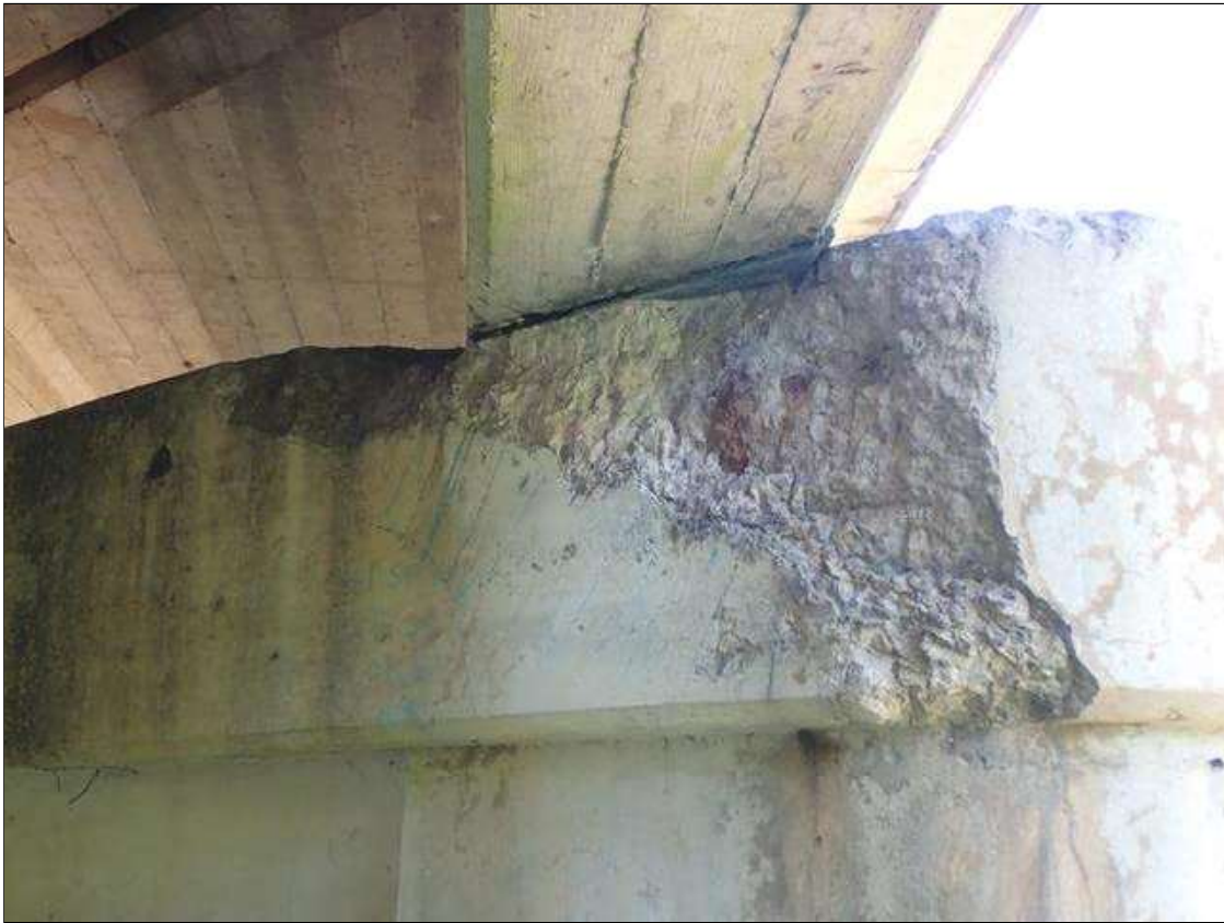
Bent 1 Cap 1: [PAR] SOUTH FACE AT GIRDER 4, SPALLING WITH EXPOSED REBAR [5' x up to full height x up to 8' deep] WITH APPROXIMATELY 20% LOSS OF BEARING AREA, NO MEASURABLE SECTION LOSS
