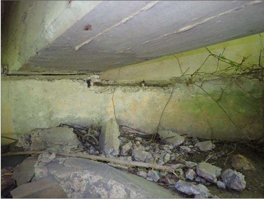
End Bent 1 Cap 1: [PAR] LEFT OUTBOARD END AT THE TOP EXTENDING TO GIRDER 1, SPALLING WITH EXPOSED REBAR, DELAMINATION AND HORIZONTAL CRACKING TO 1/4" WIDE [APPROXIMATELY 3' LONG X UP TO 1' WIDE X UP TO 3" DEEP] WITH FLAKING RUST AND PITTING UP TO 1/16" DEEP, APPROXIMATELY 5% LOSS OF BEARING AREA
