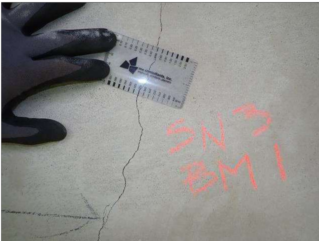
Span 3 Beam 1: along exterior face multiple vertical and diagonal cracks (full height x 0.02")
