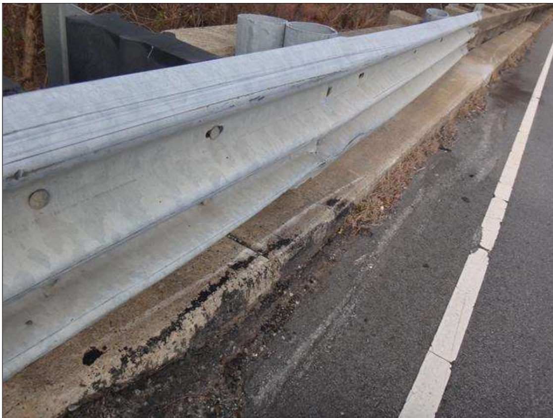
southwest guardrail at end bent 1, impact damage (6ft)
