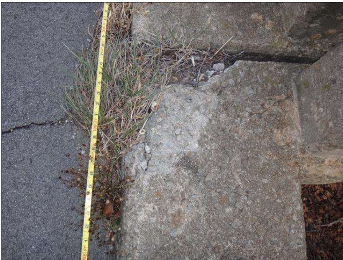
Span 5 Right Bridge Rail: 14" x 13" x 2 1/2" deep spall with exposed rebar with no measurable section loss in curb at pier 5.
