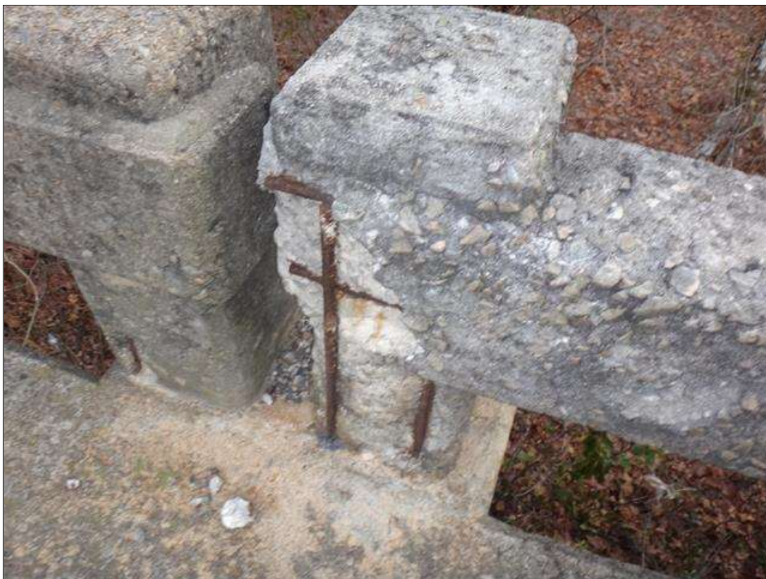
Span 7 Right Bridge Rail: Post #3, Spall with Exposed Steel with Section Loss in rebar 3/8" Remaining, (1.5' high x 9" wide x 2" deep.)
