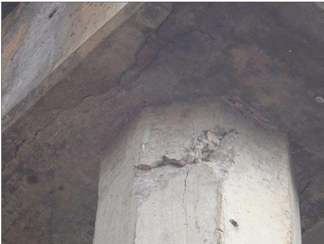
Bent 3 Pile 1: top of pile, west face, Spall no exposed steel, (8" h. x 10" wide. x 1" deep.)
