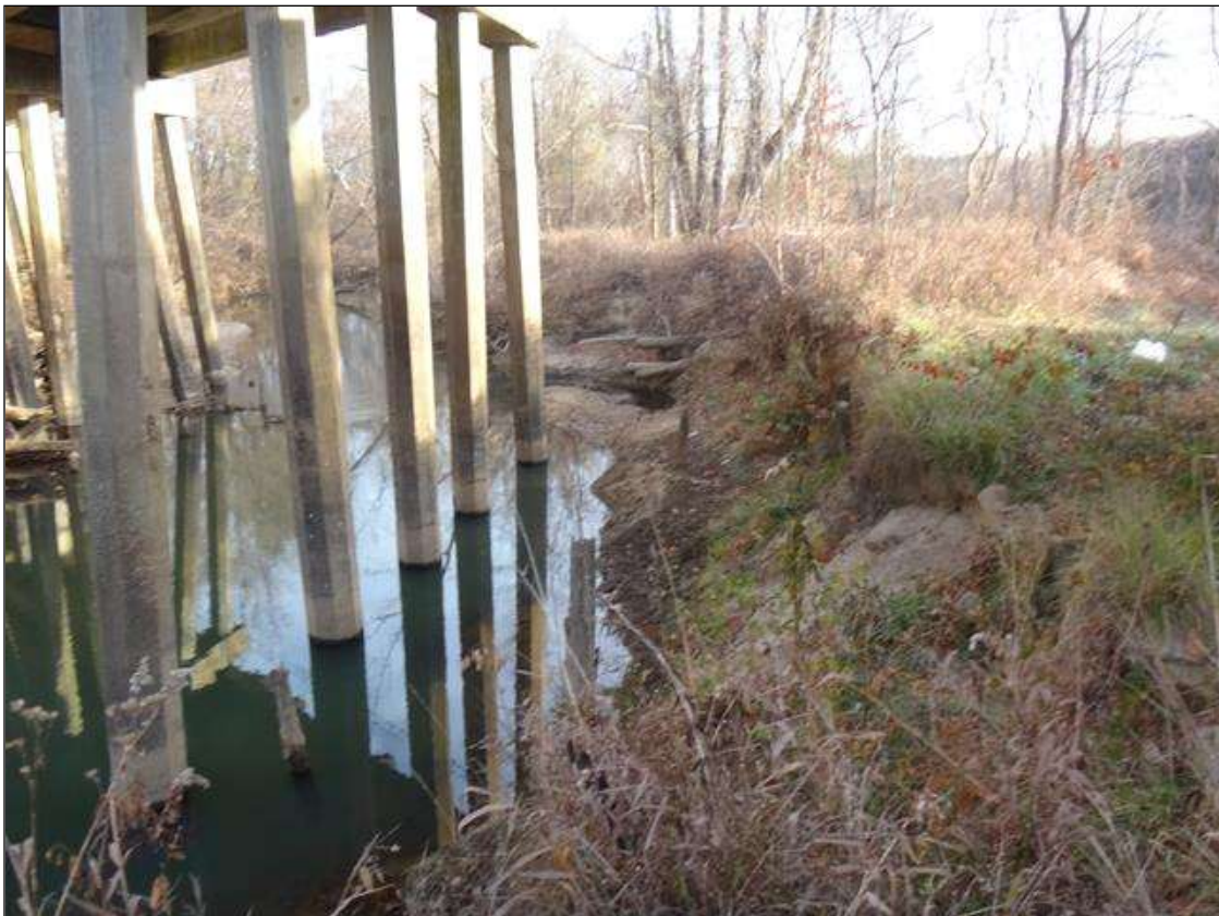
south streambank at bent, scour (75ft x 10ft x 8ft)
