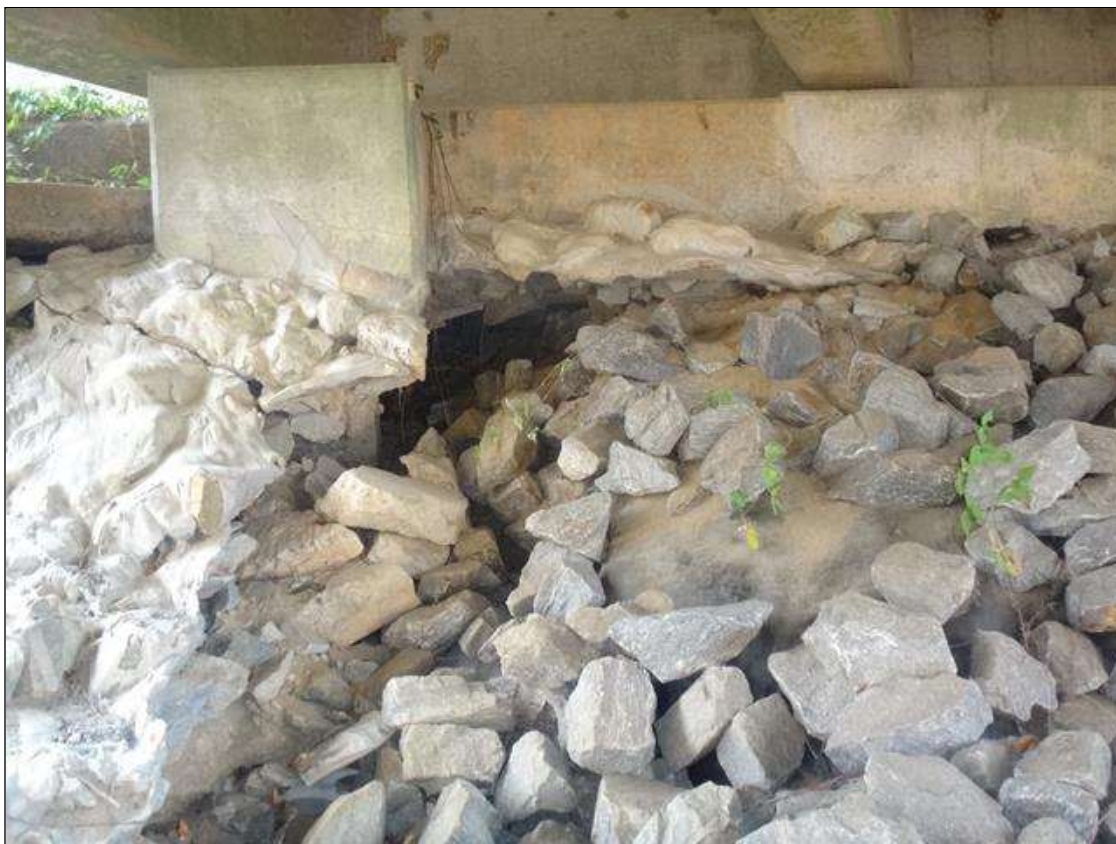
(PAR) end slope protection east end, erosion (10ft x 5ft x up to 2ft) undermining cap (up to 4ft) (photo 2 of 2)
