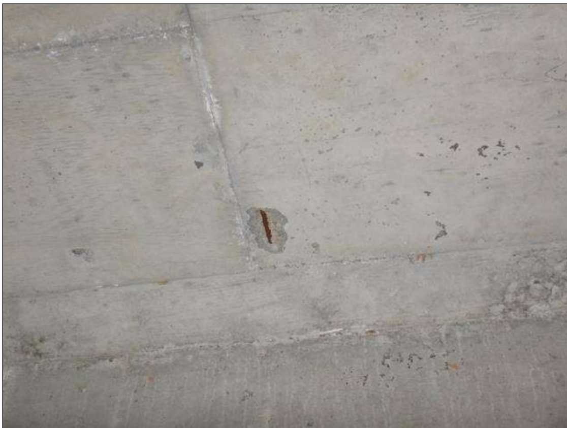
Span 1 Deck: Bottom of deck, bay 3, 12' from End Bent 1, Spall with Exposed Steel, no Section Loss in rebar, (5" x 3" x 1/2" deep.)
