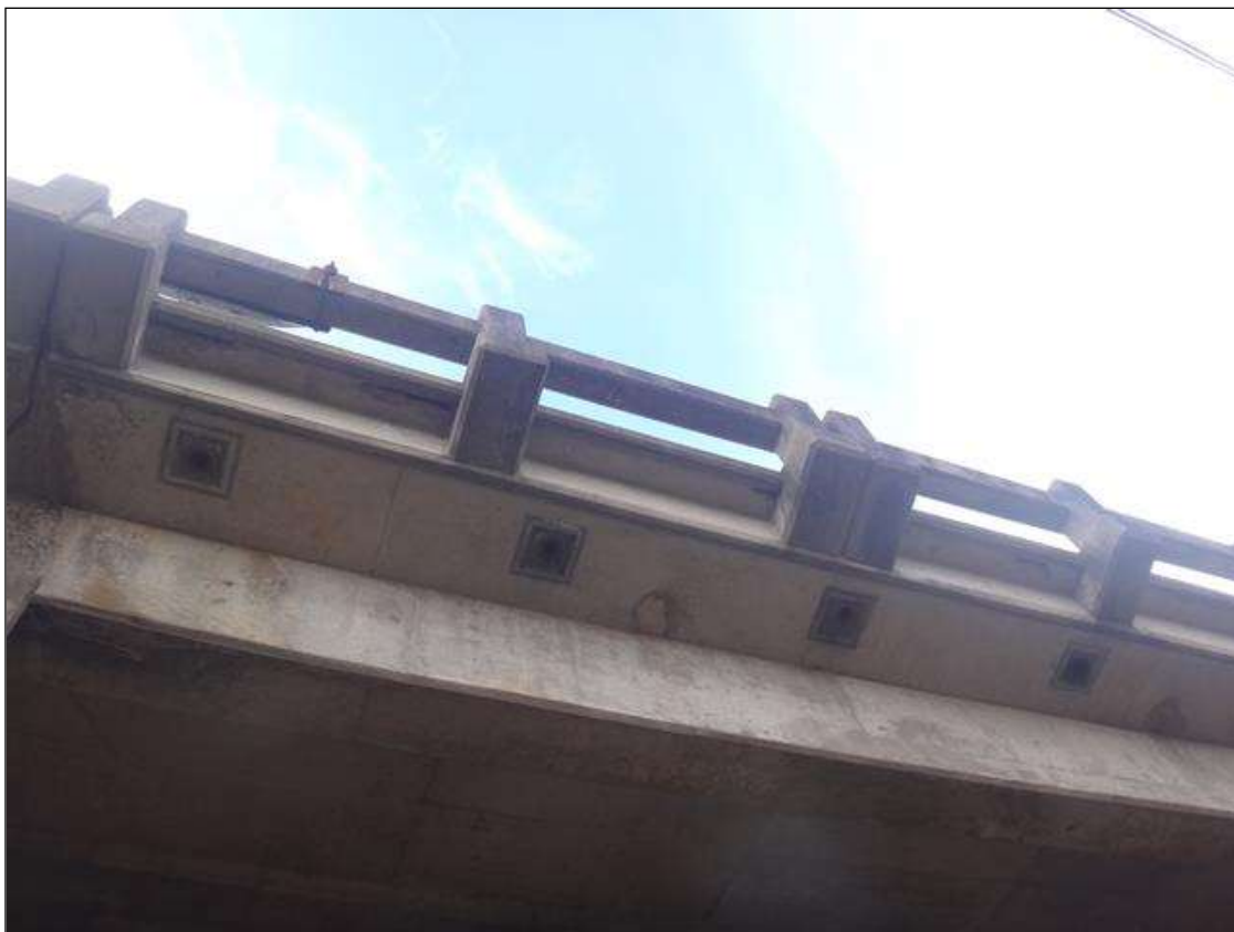
Span 2 Deck: Bottom of deck, East overhang near Bent 1,(4) spalls with exposed rebar, no Section Loss, (2' long x 4" wide. x 1" deep.)
