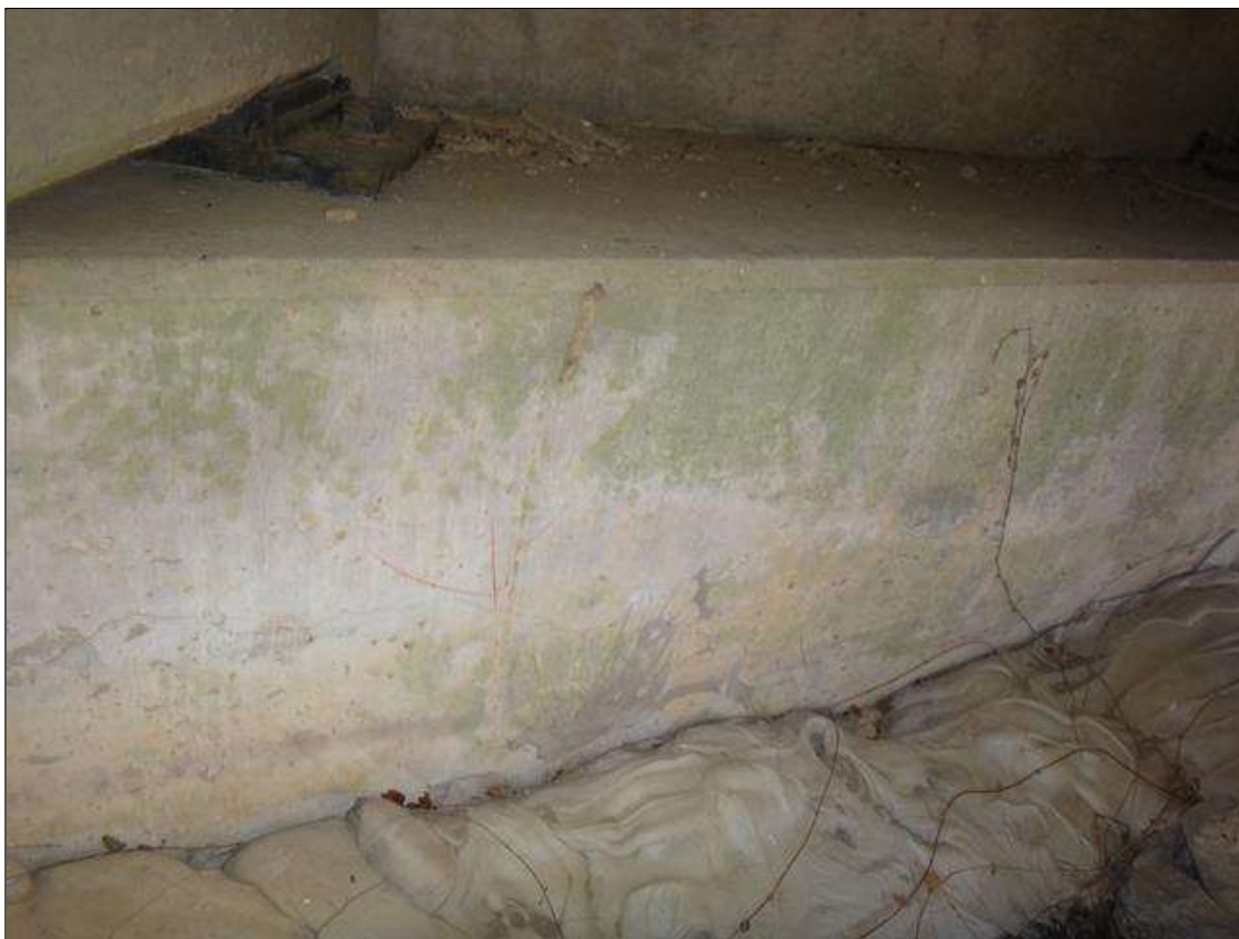
End Bent 1 Cap 1: 1/32" horizontal cracking 20' long in front face of cap under beams 1-3.
