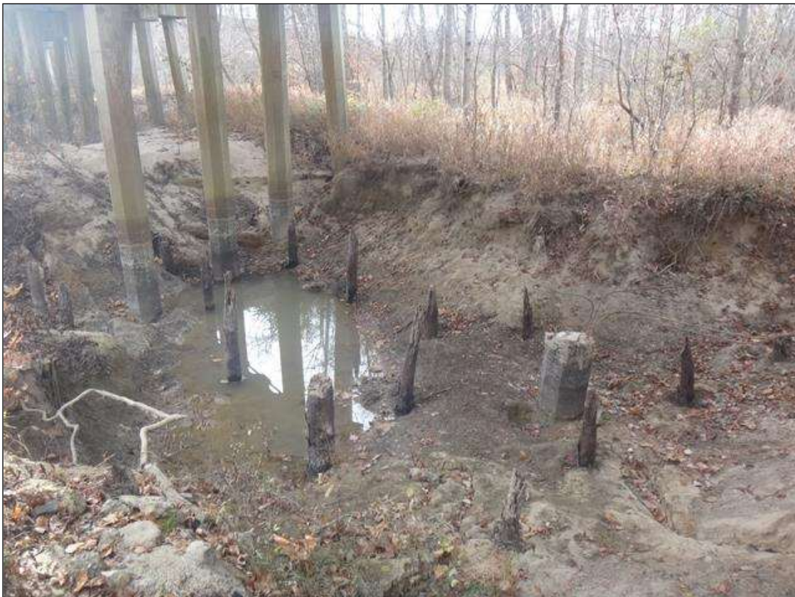
Scour: Span 6, scour hole (full length x full width x up to 9ft)
