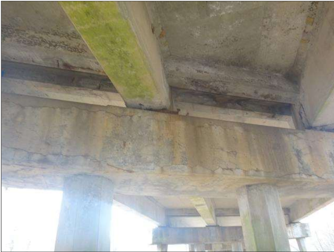
Bent 6 Cap 1: 1/8" horizontal cracks up to 25' long near top and bottom of north and south faces of cap, with rust staining. Bottom of cap, between piles 4 and 5, cracking 1/16" wide with rust staining and efflorescence.
