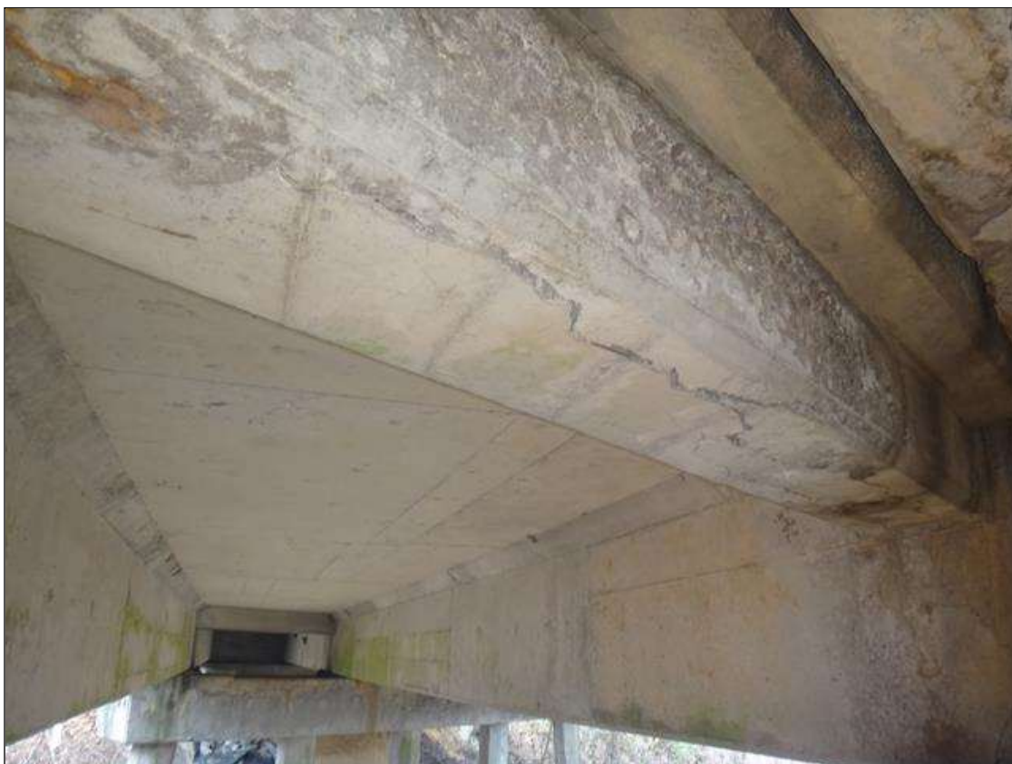
end diaphragm at bay 3 at bent 4, multiple longitudinal cracks with rust staining (full length x up to 1/8in)
