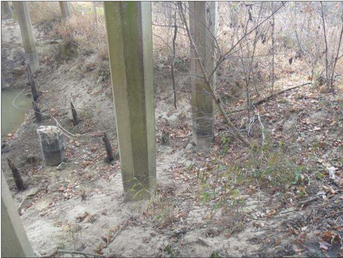
Bent 6 Pile 1: from pile 1 to 3, scour/erosion (15ft x up to 7ft)
