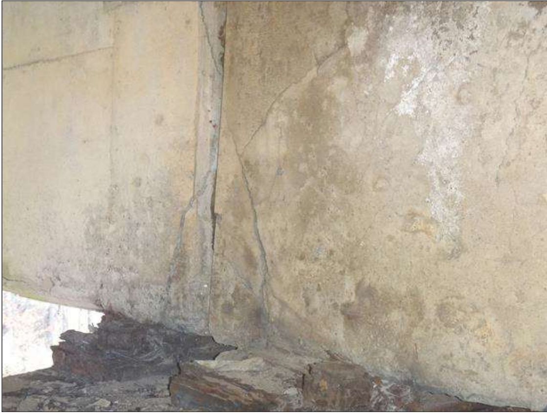
Span 7 Beam 2: at pier 6, east face, cracking 1/8" wide and Delamination (12" x full height) and Spall with Exposed Steel with Section Loss 1/16" deep (3' high x 1' long x 1-1/2" deep,) spall wraps around under bottom of girder (1' wide x 1' long x 1" deep.)
