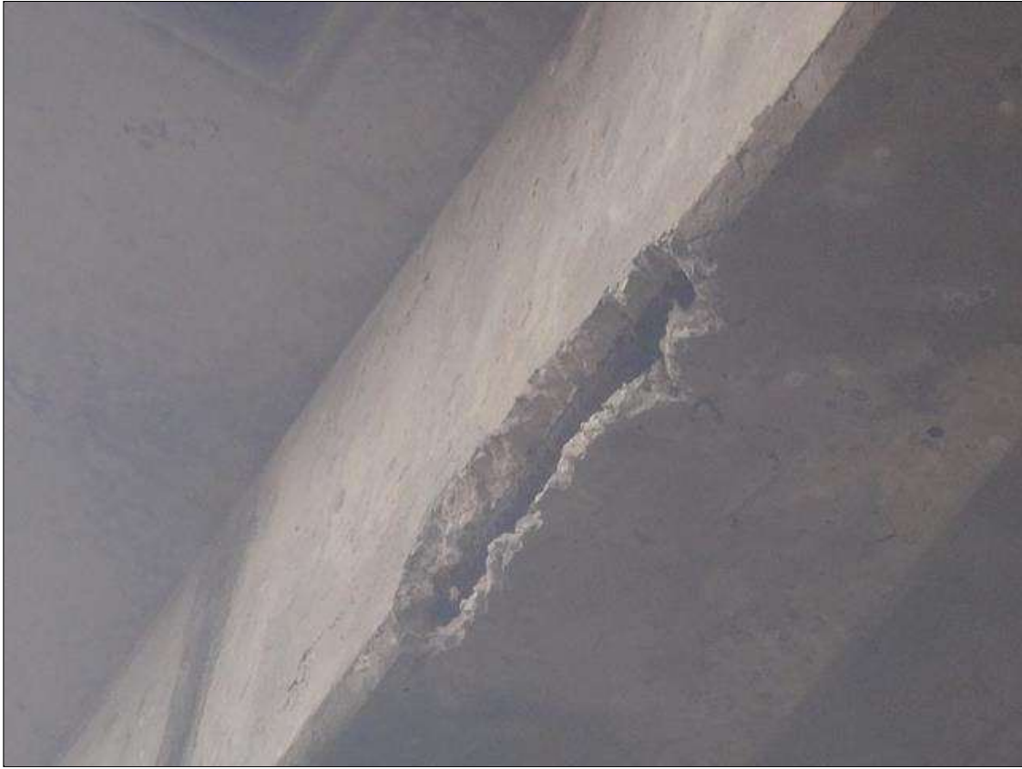
Span 3 Beam 4: (PAR) 3' long x 4" wide x 1" deep spall with exposed rebar with no measurable section loss at mid span bottom east corner.
