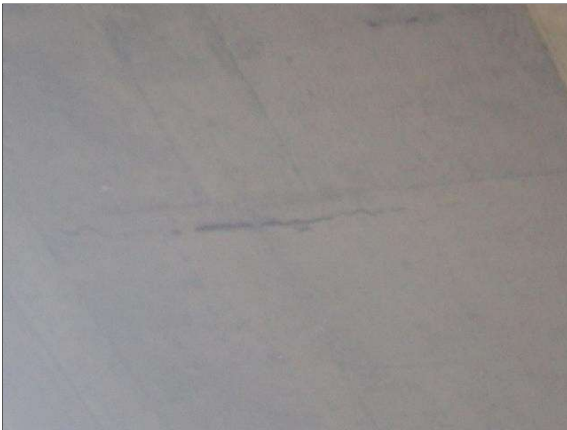
Span 3 Deck: bay 3 underside 15ft from bent 2, spall/delamination (6ft x 2in x 1/2in) with exposed rusted rebar
