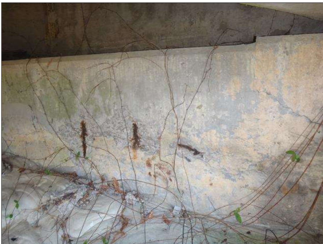
End Bent 1 Cap 1: below bay 1, Delamination/ spalling with exposed rebar, no Section Loss, (3' long x 1' high x 3/4" deep)
