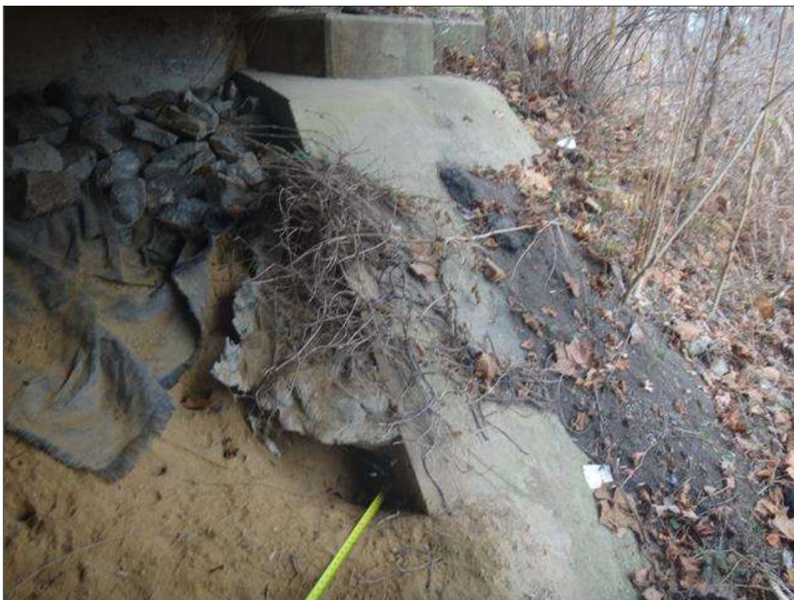
end bent 2 slope protection flume, undermining (up to 3ft x 1ft)
