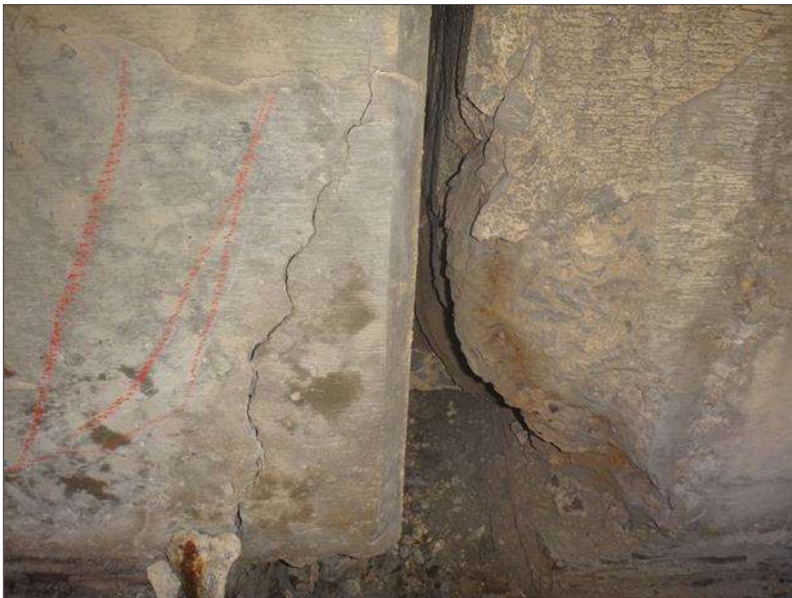
Span 6 Beam 4: at bent 6, spall (12in x 6in x 10in)
