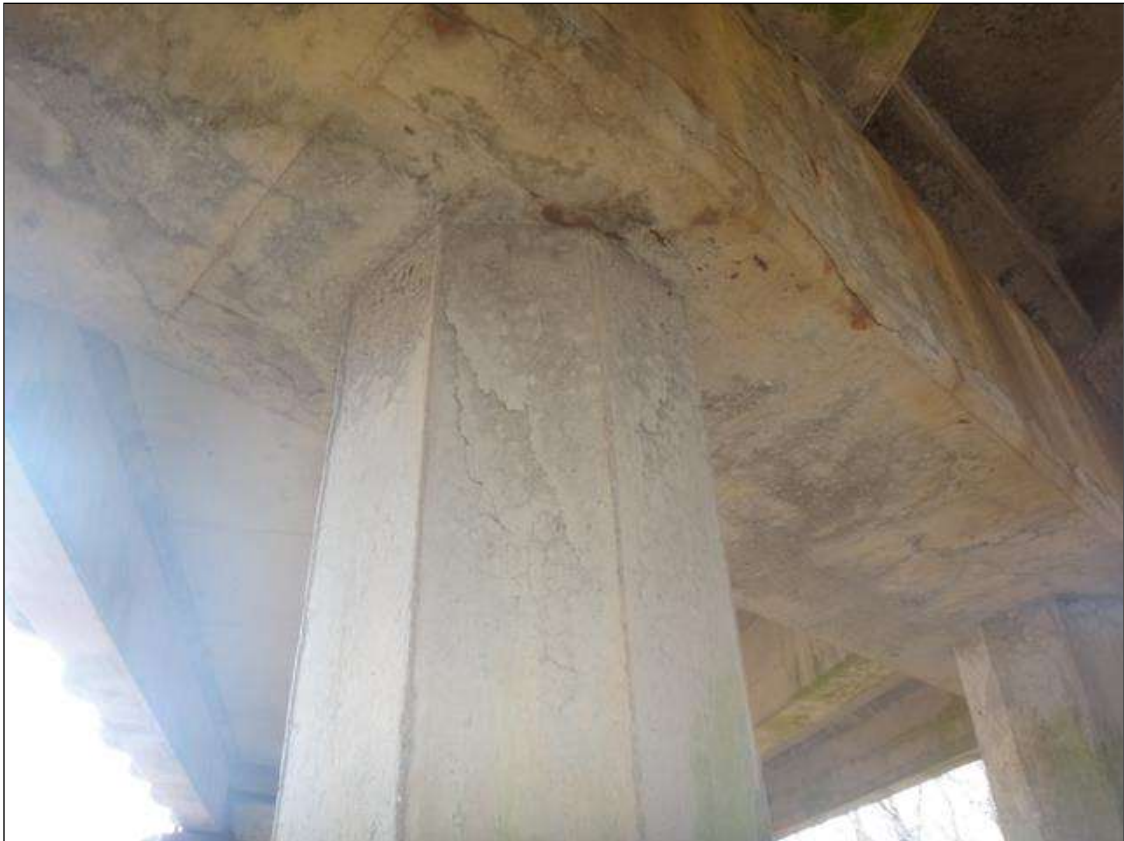
Bent 6 Pile 4: top of pile, north side, Delamination (12" h. x 8" wide.)
