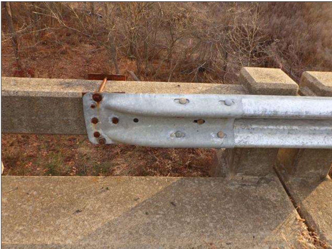
southeast guardrail attachment (damaged area)
