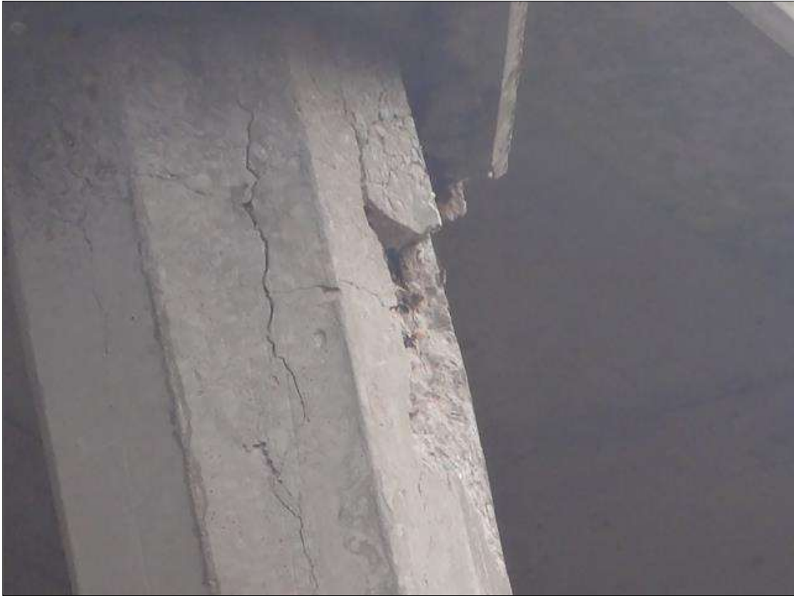
Bent 2 Pile 1: (PAR) west/south faces of column starting at bottom of cap, 5' long x 20" wide area of delamination with cracks up to 1/8" wide and a 2' high x 10" wide x 1.5" deep spall with exposed rebar with section loss 1/8" deep. (photo 1 of 2)
