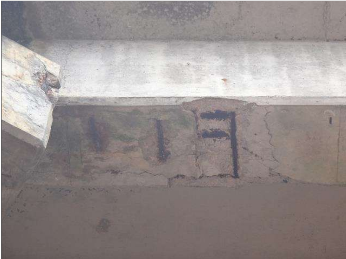
Span 5 Beam 4: (PAR) at pier 4, (5' long x 1.5' wide x 4" deep,) area of Delamination/ Spall with exposed rebar with section loss 1/8" deep.
