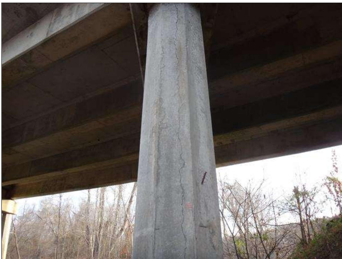
Bent 1 Pile 1: 1/32" vertical/horizontal cracks up to full height on south and north faces of column starting at bottom of cap.
