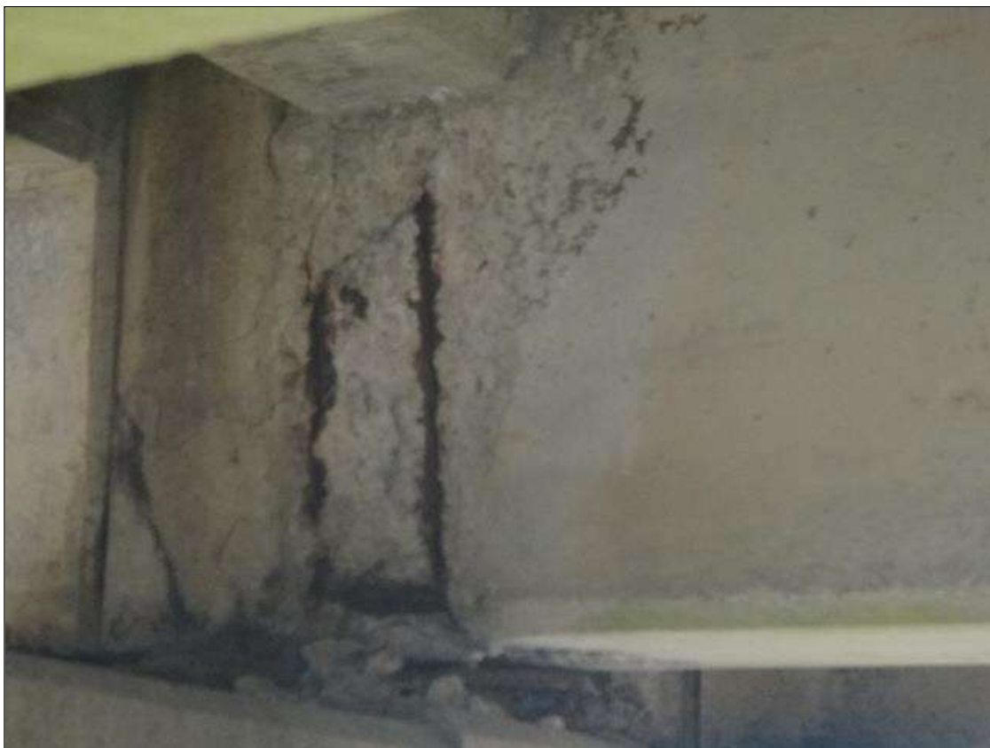
Span 6 Beam 1: (PAR) at pier 6, 3' long x 1.5' wide x 3" deep Delamination/ spall with exposed reinforcing with minor section loss up to 1/8" deep on bottom of girder.
