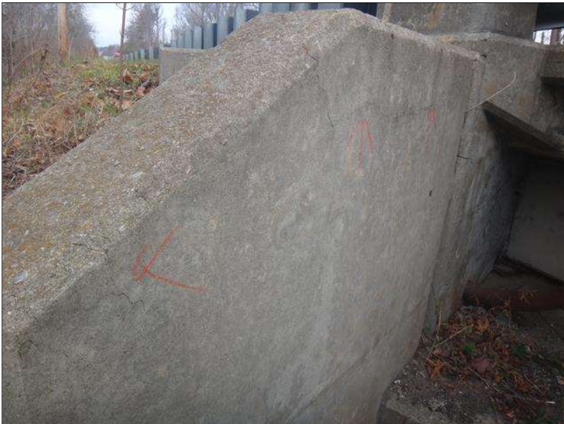
southeast wingwall, horizontal and vertical cracks (up to 2ft x 1/32in)
