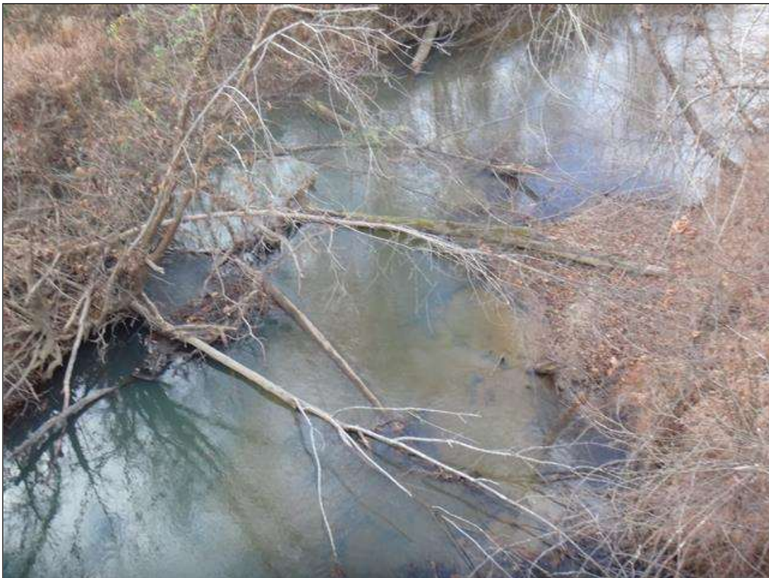
75ft upstream, multiple trees blocking waterway
