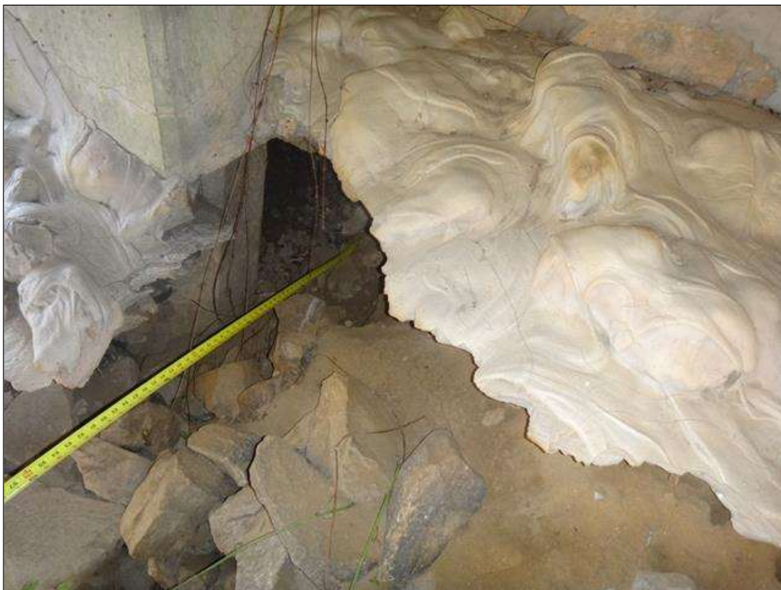
(PAR) end slope protection east end, erosion (10ft x 5ft x up to 2ft) undermining cap (up to 4ft) (photo 1 of 2)
