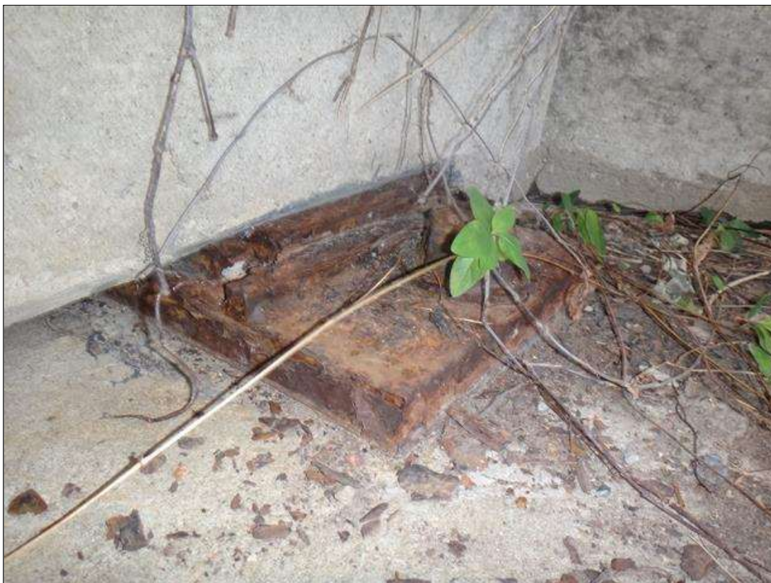
Span 1 Beam 1 - Near Bearing: Active Corrosion and Section Loss up to 1/16" deep, in plates.
