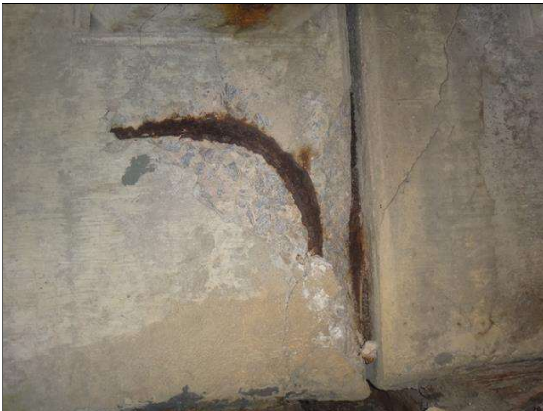
Span 2 Beam 3: over pier 1, west face of girder, Spall with exposed rebar with no measurable section loss (12" x 8" x 1" deep,) and Delamination (12" h. x 5" long x 2" deep.)
