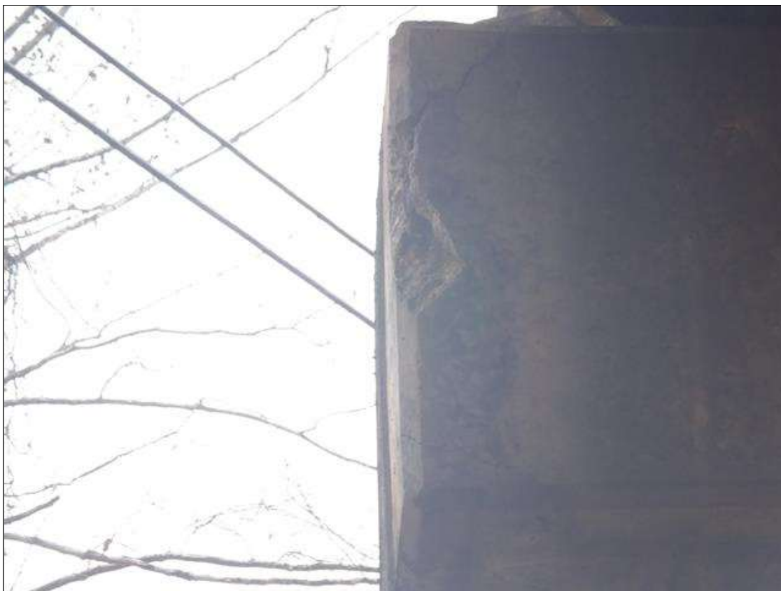
Bent 4 Cap 1: on northeast corner, no measurable section loss, (12" high x 6" wide x 1-1/2" deep,) and Delamination 6" x 6" x 7".
