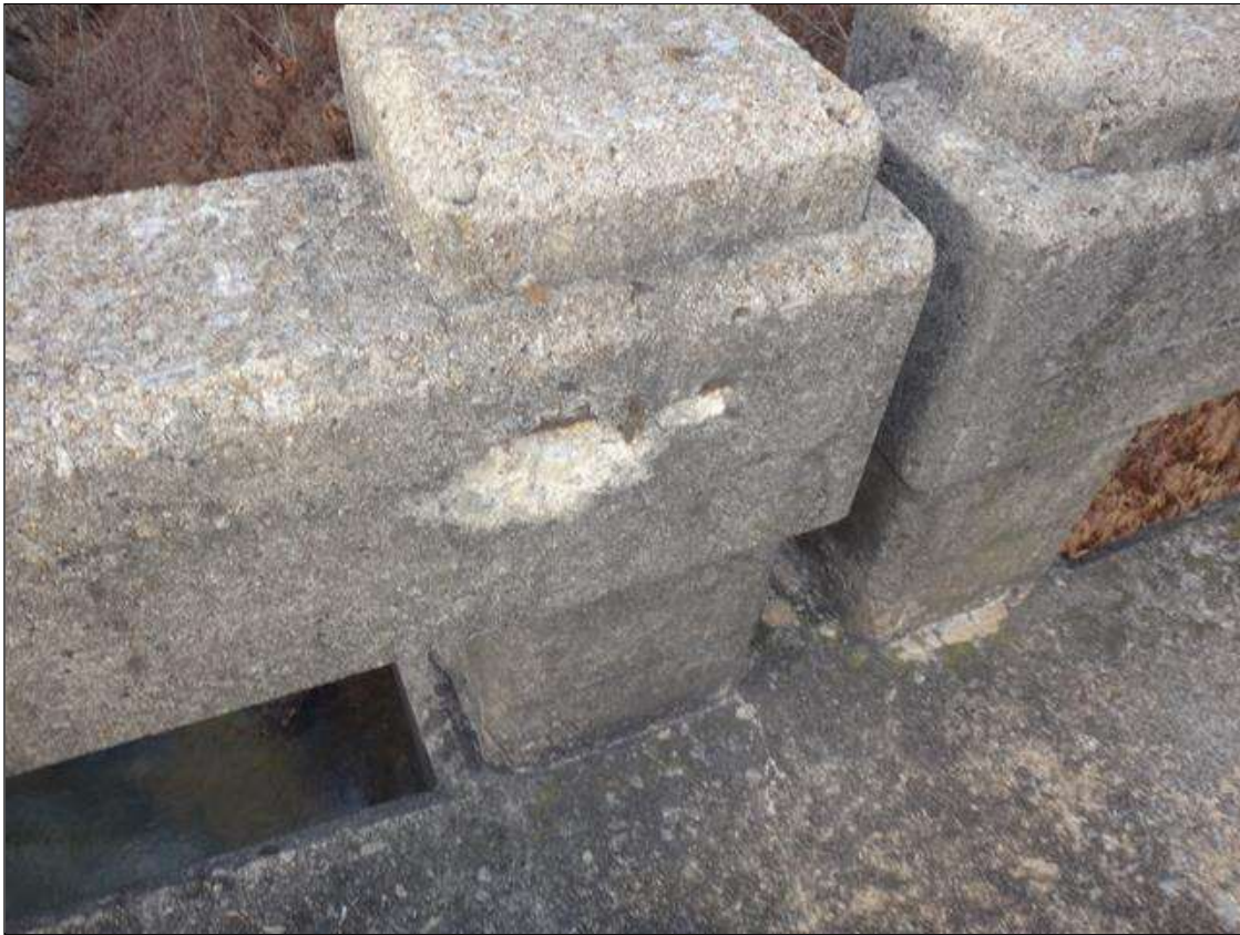
Span 3 Left Bridge Rail: 6" x 3" x 1" deep spall with exposed rebar with no measurable section loss in rail at Post 6.
