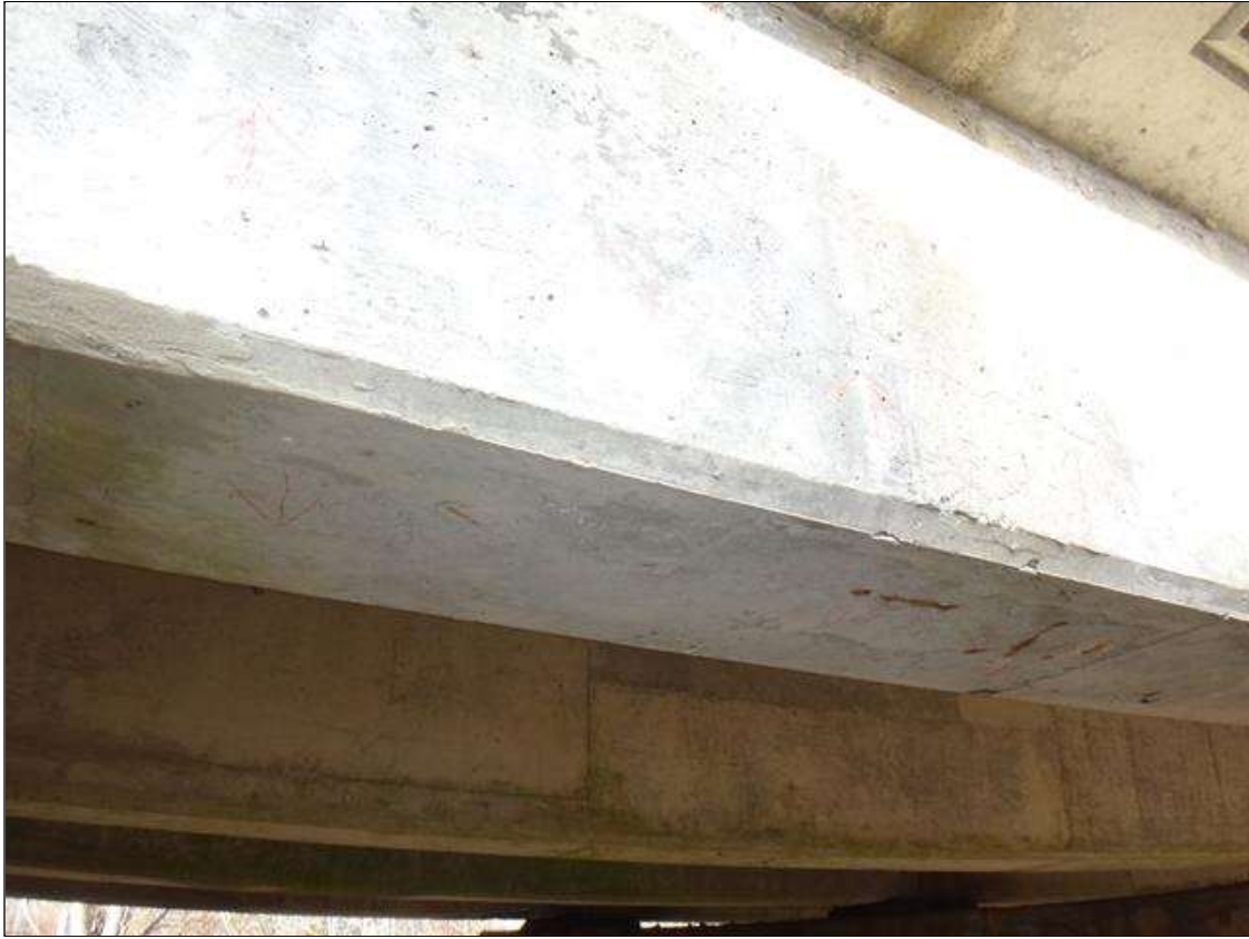
Span 1 Beam 4: underside and east face near end bent 1, multiple longitudinal and horizontal cracks ( up to 6ft x 1/32in)
