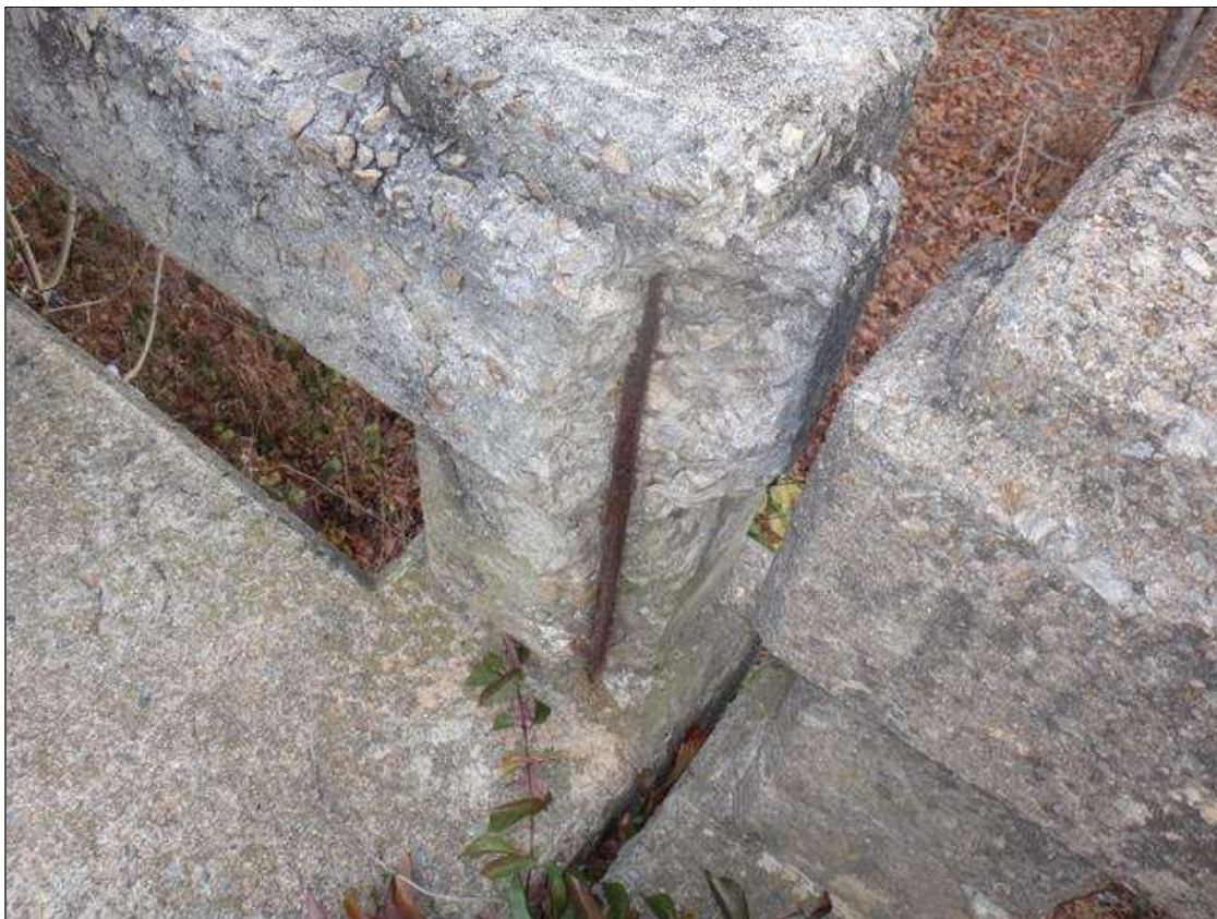
Span 7 Right Bridge Rail: 2' high x 4" x 2" deep spall with exposed rebar with no measurable section loss in rail post at pier 6.
