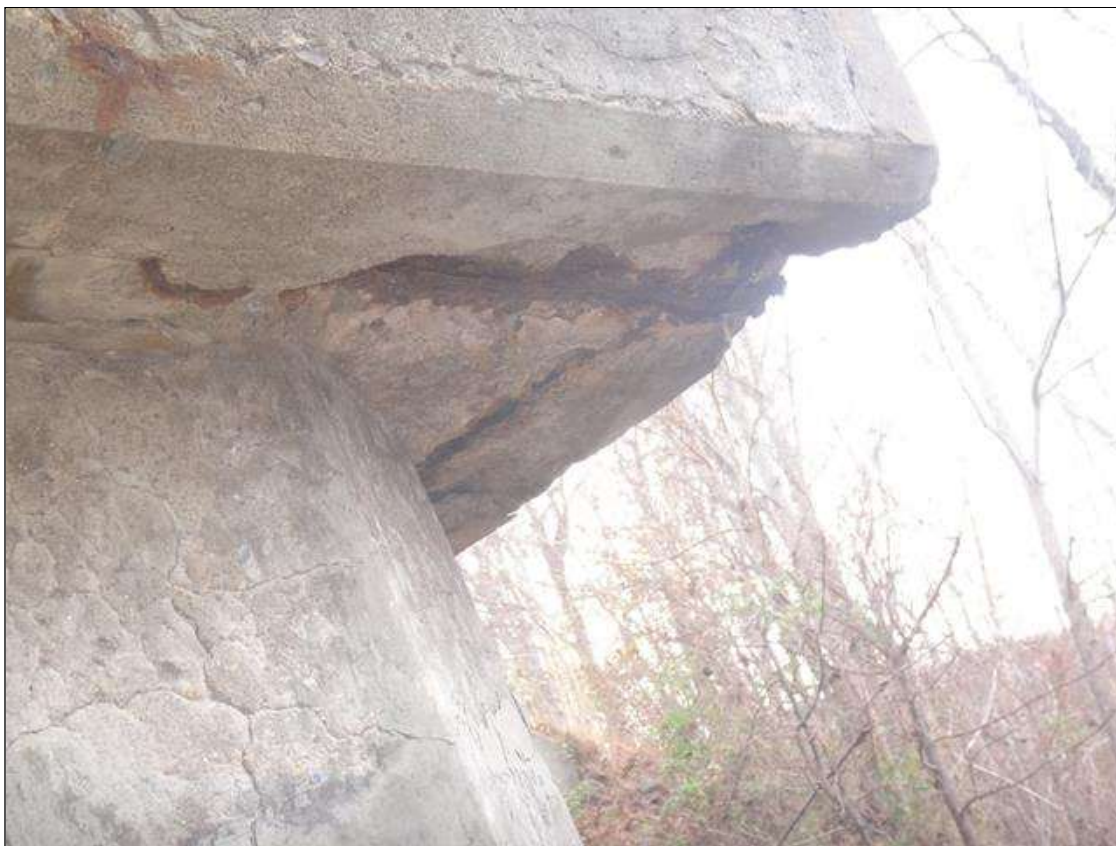
Bent 1 Cap 1: 4" diameter spall 1/4" deep in bottom of cap bay 1 at column 1.
