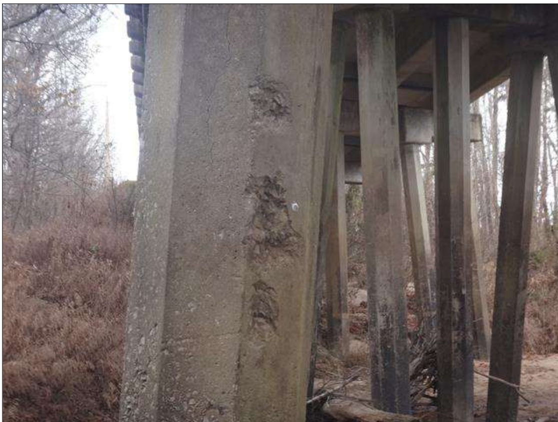
Bent 2 Pile 1: south face near mid height, multiple spalls (up to 8in diameter x 1in)
