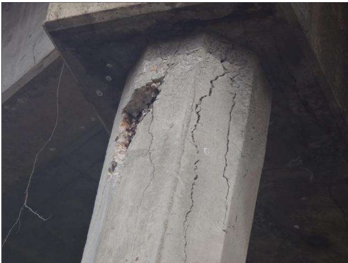
Bent 2 Pile 1: (PAR) west/south faces of column starting at bottom of cap, 5' long x 20" wide area of delamination with cracks up to 1/8" wide and a 2' high x 10" wide x 1.5" deep spall with exposed rebar with section loss 1/8" deep. (photo 2 of 2)
