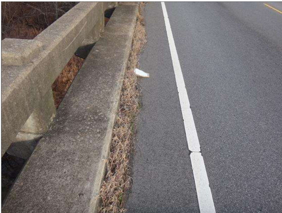
west shoulder, debris accumulation/vegetation growth (full length x 1ft) partially blocking drains
