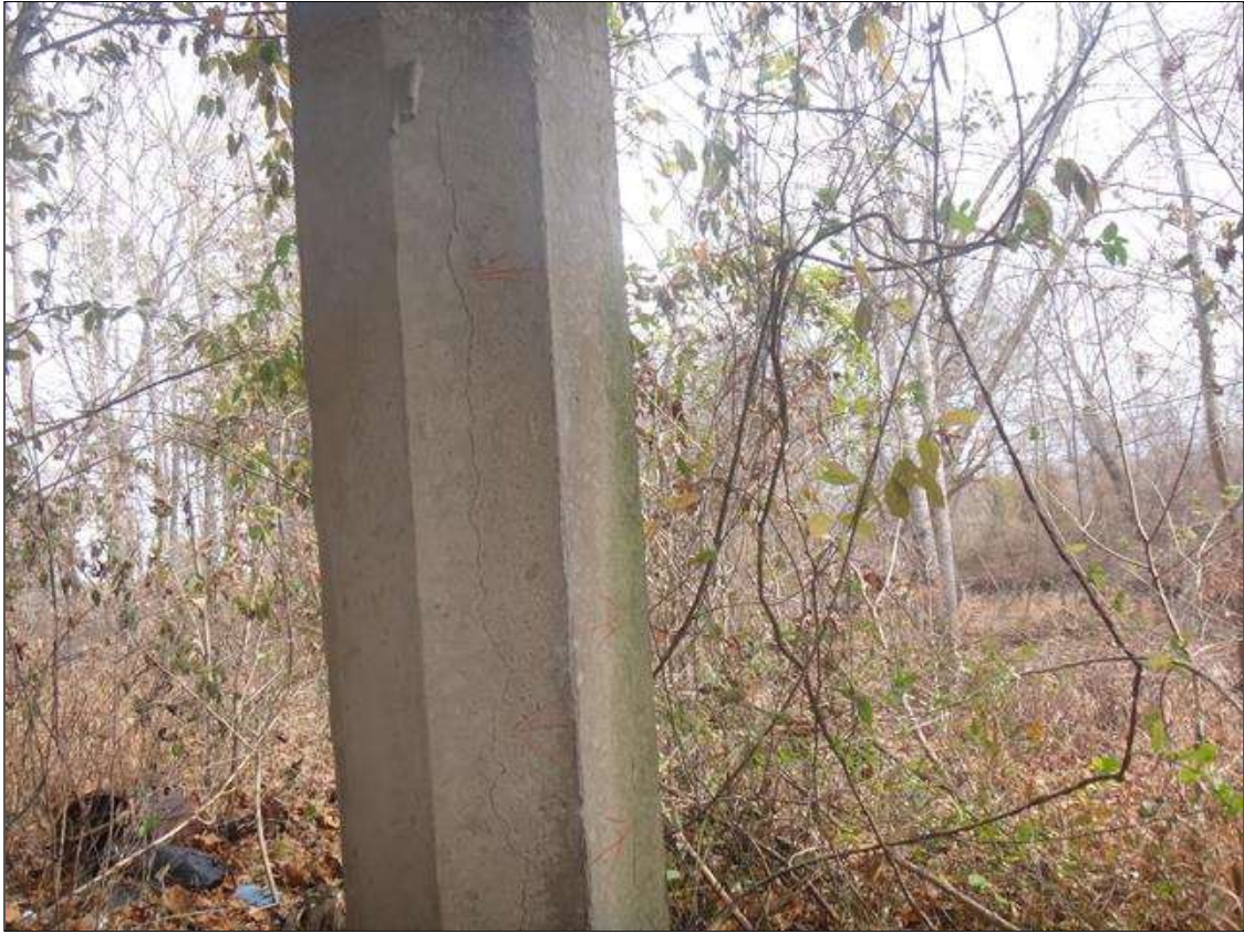
Bent 6 Pile 5: all faces, multiple vertical cracks (full height x up to 1/16in)
