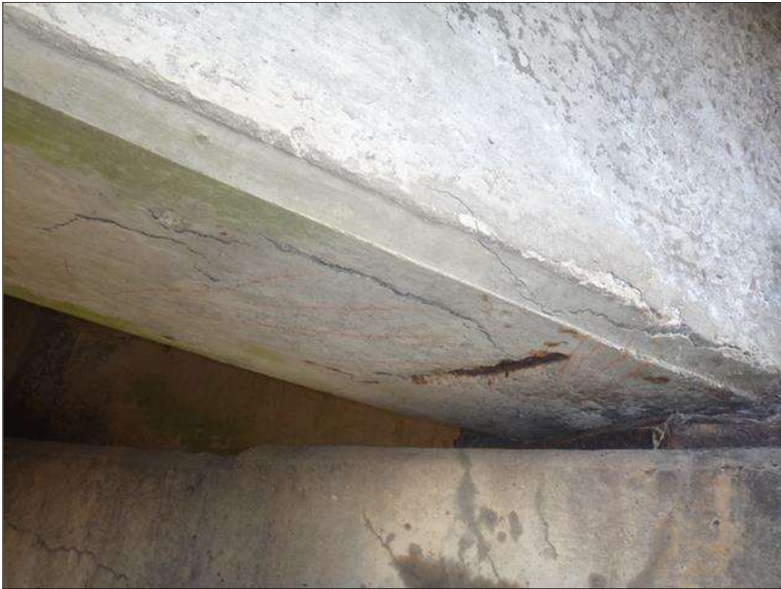
Span 6 Beam 4: 2' high x 2' wide delamination on west face of beam that extends 1' on bottom of beam at pier 5.
