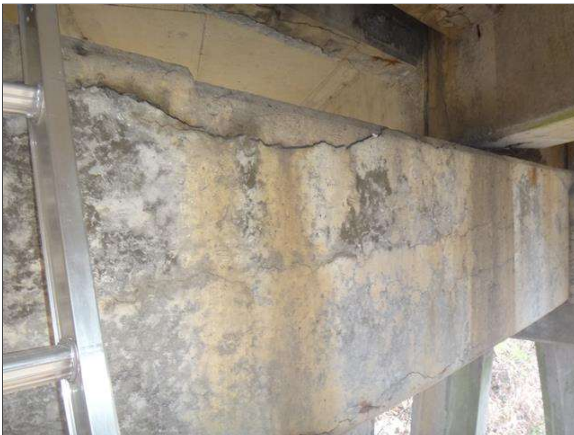
Bent 4 Cap 1: Several 1/8" to 1/4" horizontal cracks up to 10' long scattered throughout south and north faces of cap and cross caps.
