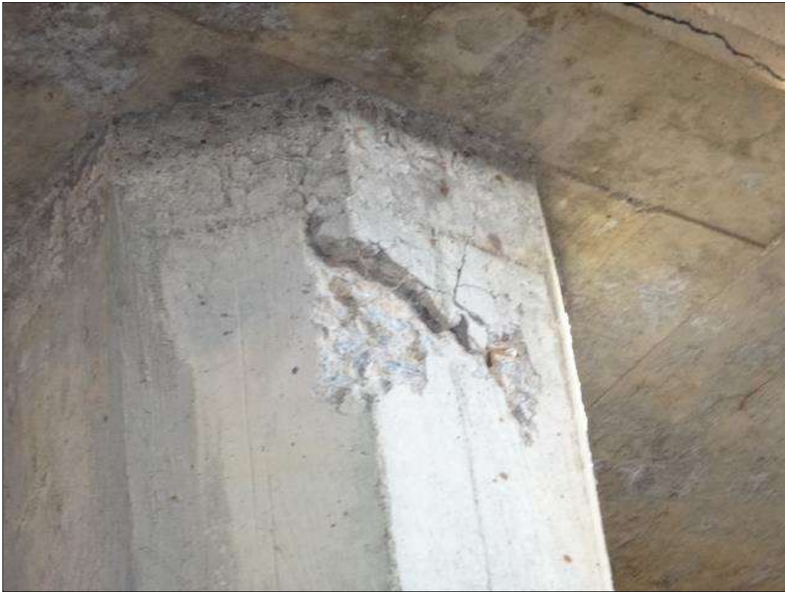
Bent 1 Pile 3: 6" high x 8" wide x 1" deep Delamination/ spall no exposed steel, at top of south face of column.
