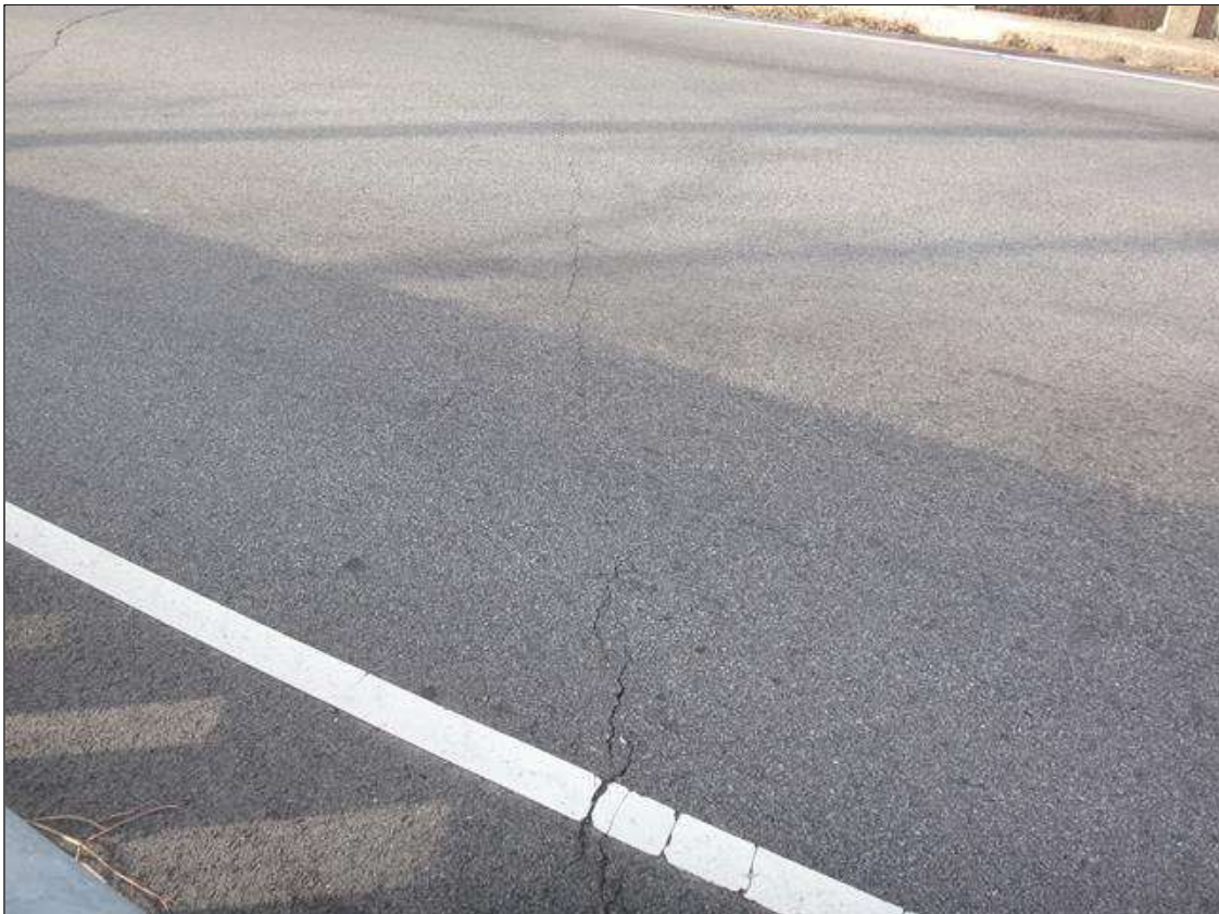
Span 1 Wearing Surface: at end bent 1, transverse crack (full width x 1/16in)
