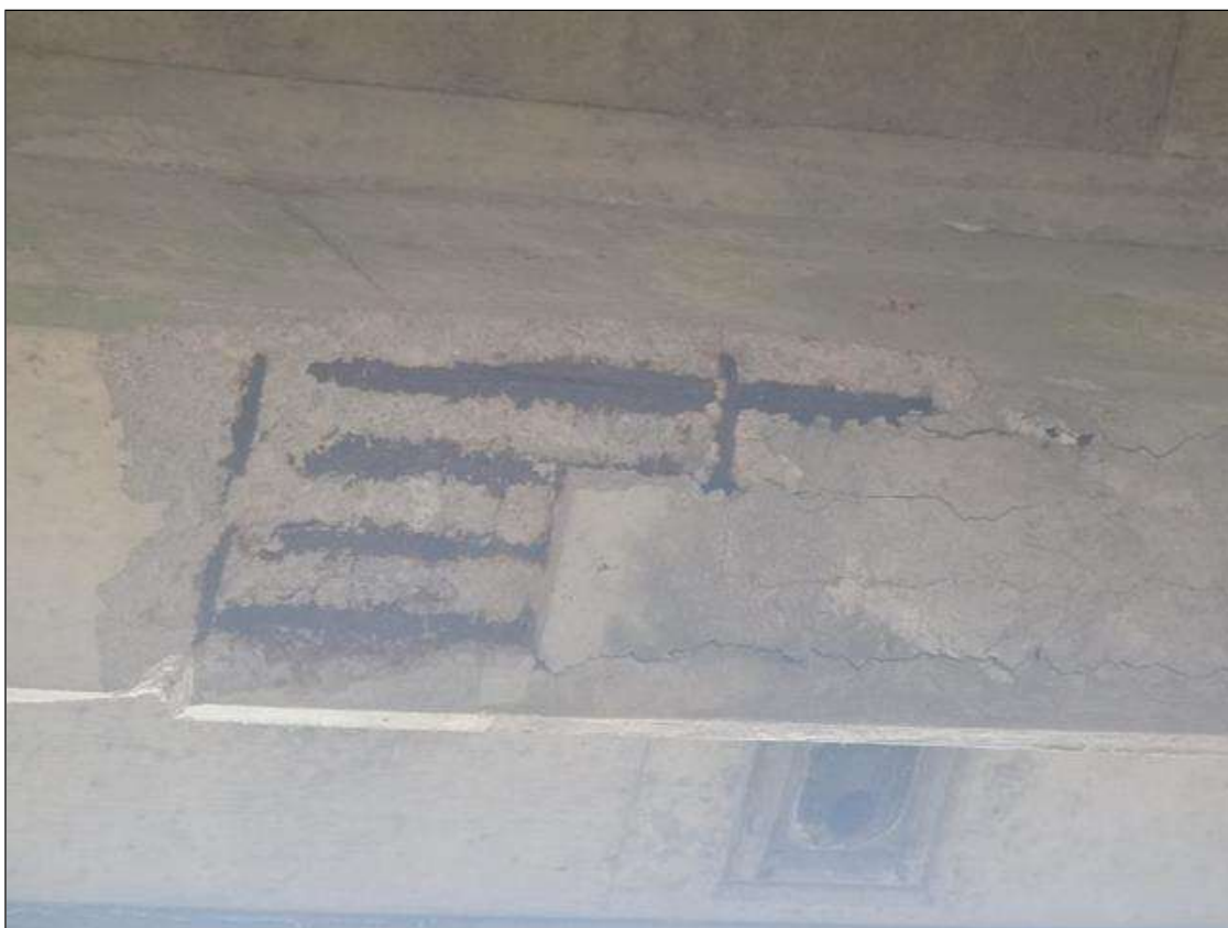
Span 2 Beam 1: (PAR) at 12' from pier 2, bottom of girder has Delamination (5' long x 1.5' wide x 2" deep,) and Spall with Exposed Steel, no measurable section loss, (30" long. x 4"h. x 2" wide.)
