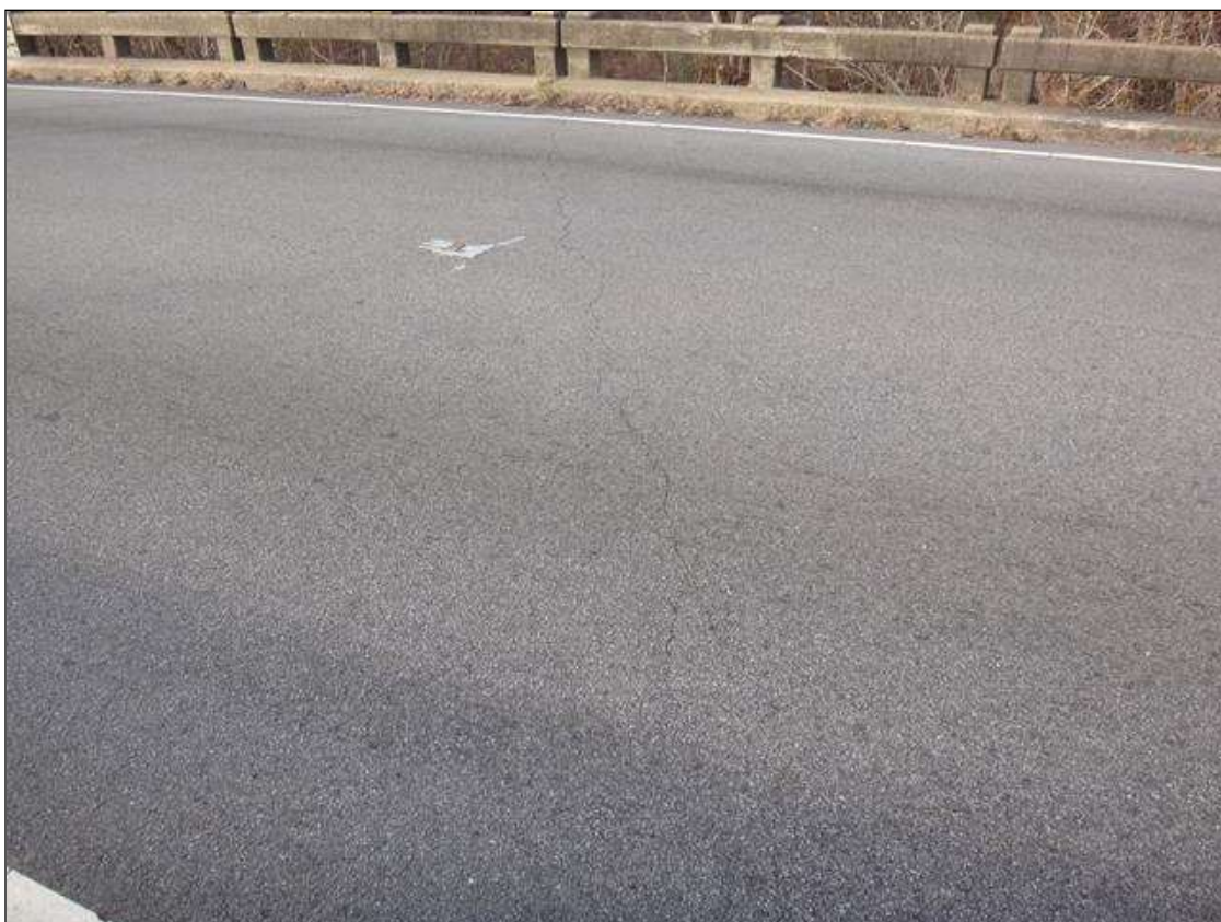
Span 2 Wearing Surface: bent 1, transverse crack (full width x 1/16in)
