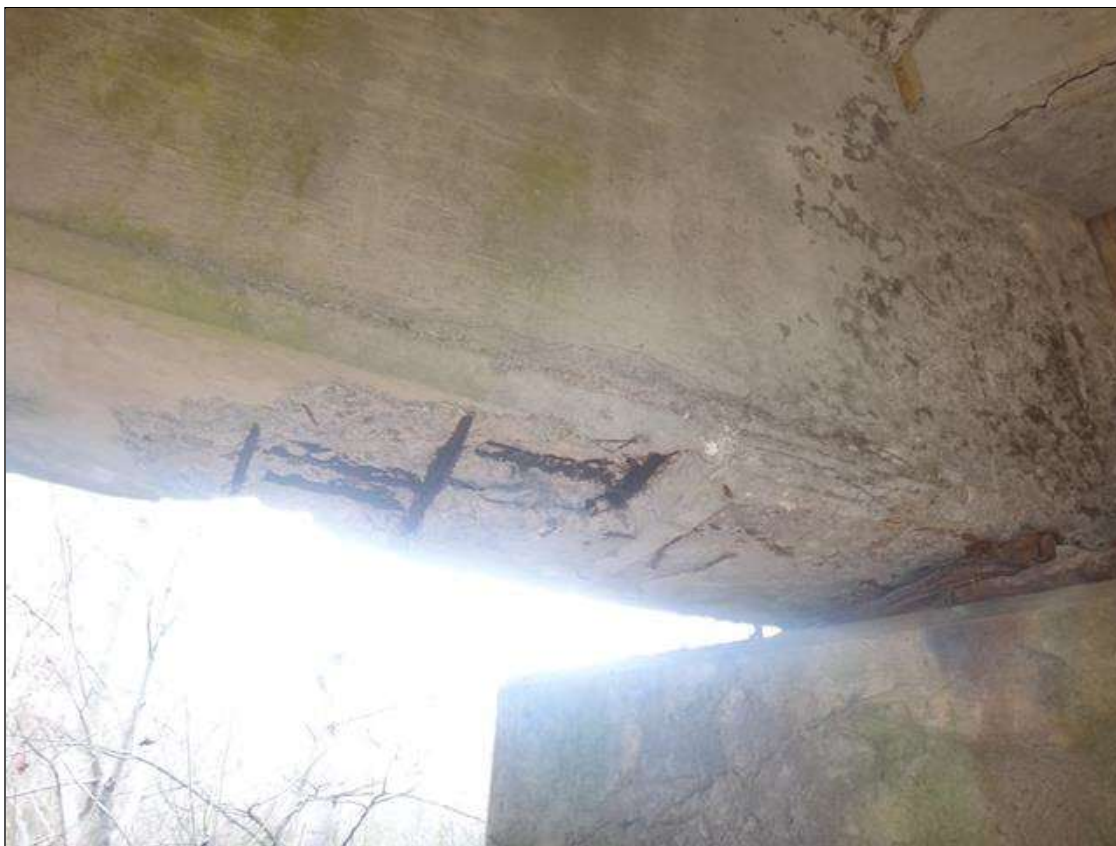
Span 5 Beam 1: (PAR) at pier 5, (3' long x 1.5' wide x 3" deep,) area of Delamination/ spall with exposed rebar with section loss 1/8" deep, on bottom of girder.
