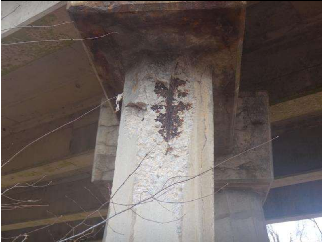
Bent 4 Pile 1: (PAR) starting at bottom of cap, West face, Spall with Exposed Steel with Section Loss 1/8" deep, (20" h. x 12" wide. x 2-1/2" deep,) South face has Delamination (5' long x 20" wide) with 1/8" wide cracking.
