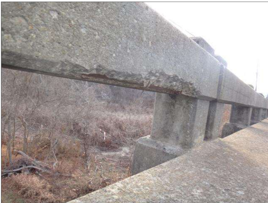
Span 2 Right Bridge Rail: 32" x 3" x 2 1/2" deep spall with exposed rebar with no measurable section loss on underside of top rail, 10' from pier 2.
