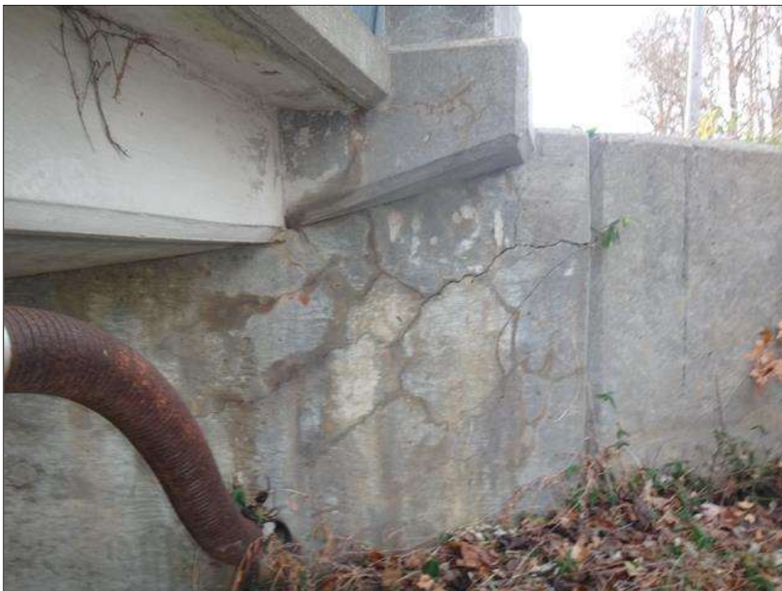
End Bent 1 Abutment: at west end of abutment, (1/16" to 1/4" wide) cracking with efflorescence.
