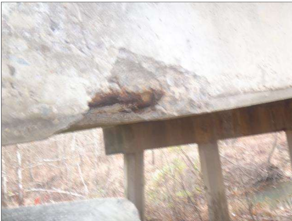
Span 5 Beam 4: (PAR) at pier 4, (5' long x 1.5' wide x 4" deep,) area of Delamination/ Spall with exposed rebar with section loss 1/8" deep. (photo 2 of 2)
