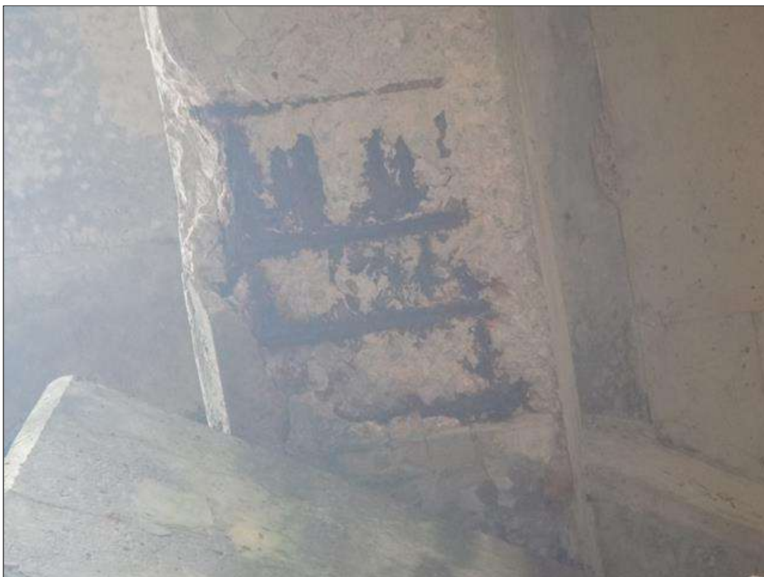
Span 5 Beam 4: (PAR) at pier 4, (5' long x 1.5' wide x 4" deep,) area of Delamination/ Spall with exposed rebar with section loss 1/8" deep. (photo 1 of 2)
