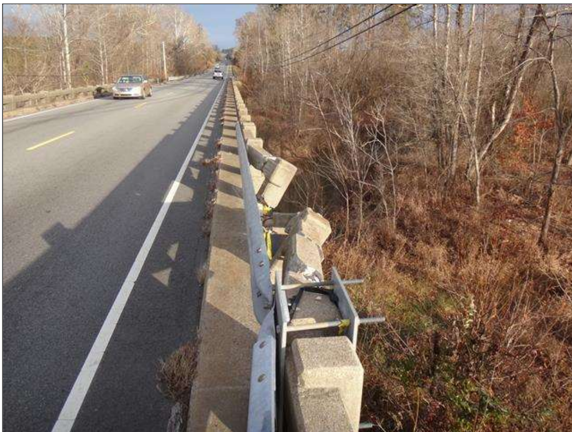
Span 1 Right Bridge Rail: (PAR) near end bent 1, impact damage (18ft) steel guardrail in place but no post
