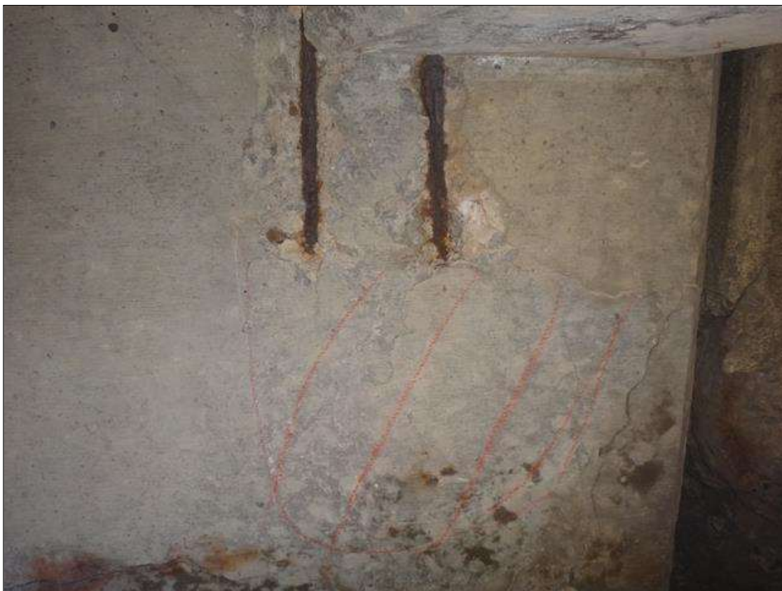
Span 7 Beam 4: 24" x 8" x 1/2" spall/delamination with exposed rebar with no measurable section loss on west face of girder at pier 6 end.
