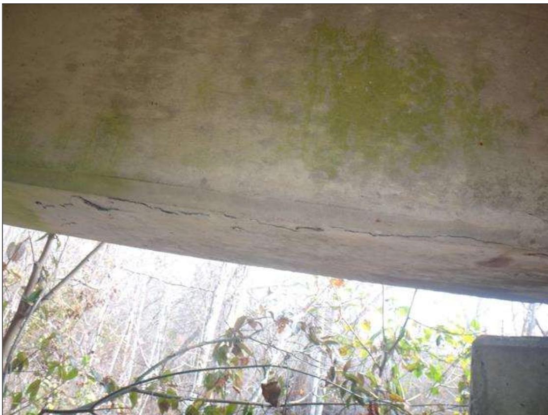
Span 7 Beam 4: underside at bent 6, delamination (3ft x full width)
