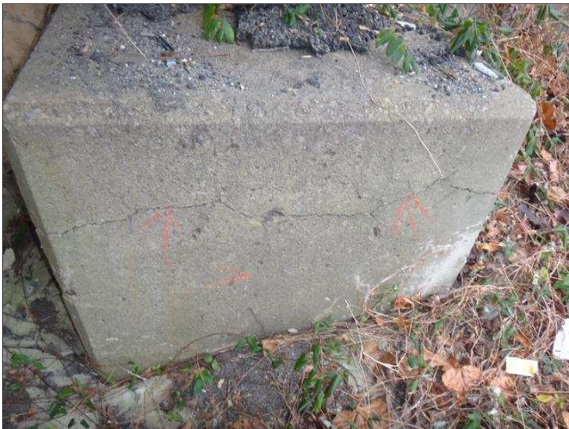
End Bent 1 Cap 1: Cap for Brace pile at west end of End Bent 1, cracks (1/16" to 1/8" wide.)
