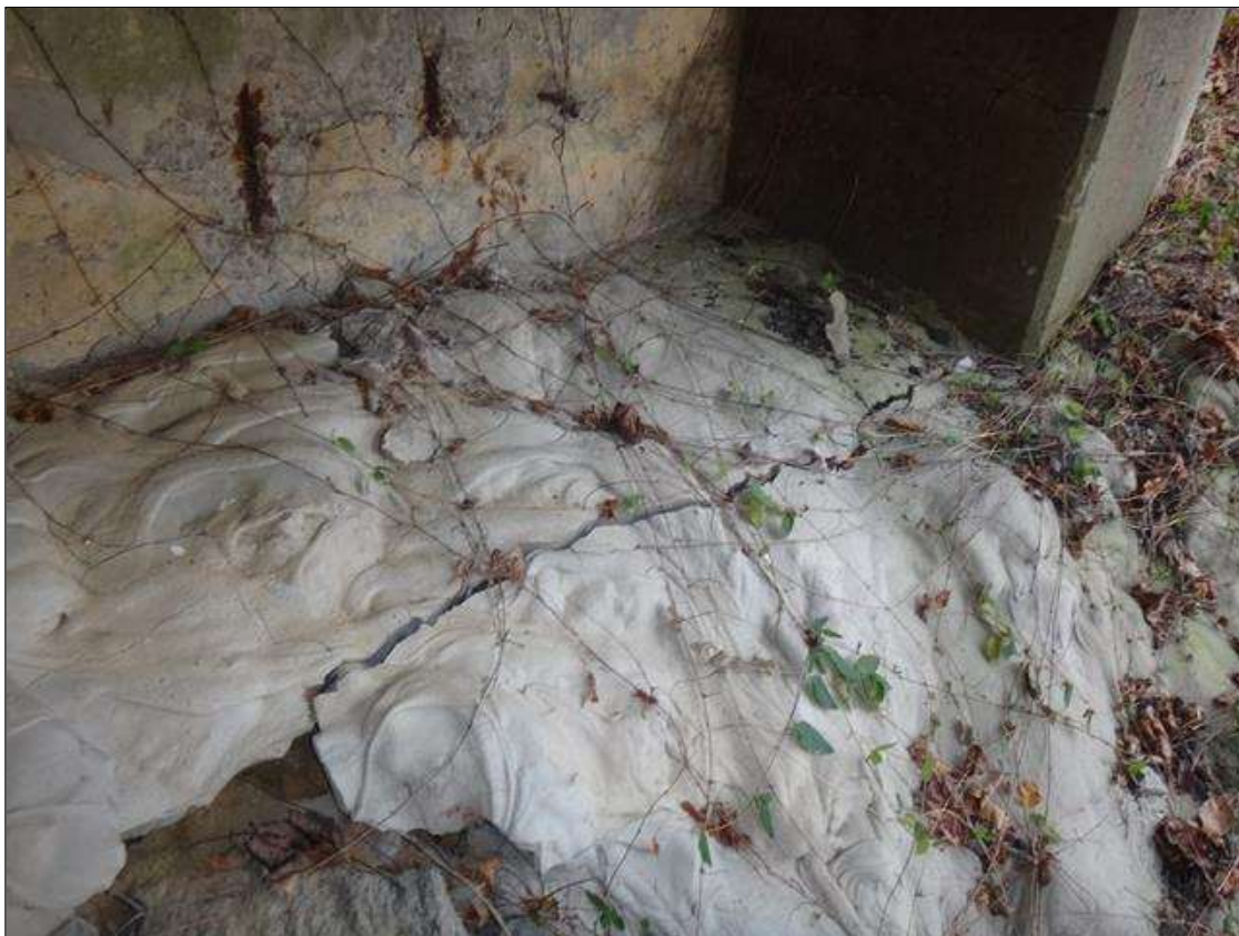
epc slope protection at west end previous repaired, transverse crack (5ft x up to 1/2in)
