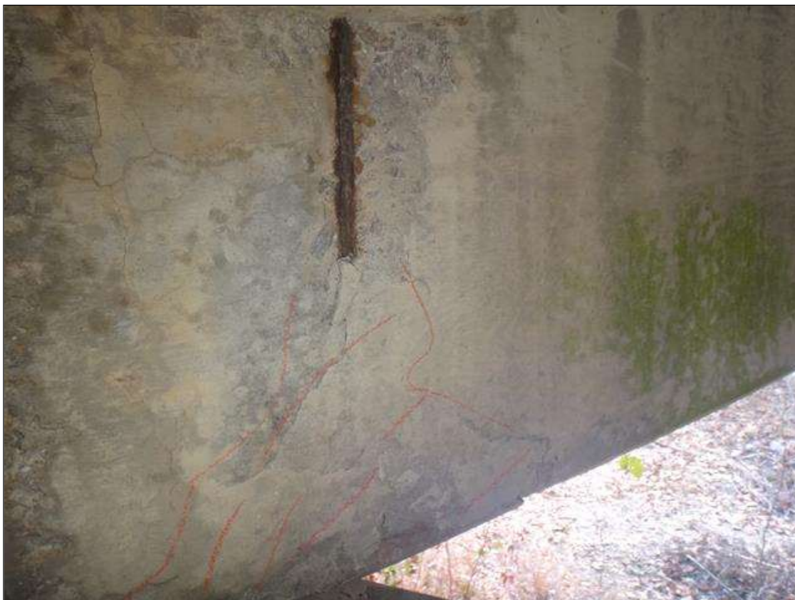
Span 6 Beam 4: west face at bent 6, spall/delamination (24in x 24in x 1/2in) with exposed rusted rebar
