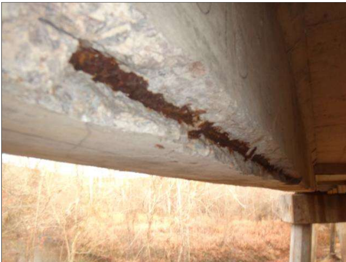
Span 1 Beam 1: PAR: at 7' from End Bent 1, bottom of girder has Delamination/ Spall with Exposed Steel with Section Loss 1/16" deep, (6'-10" x 10" wide. x 4" deep.)
