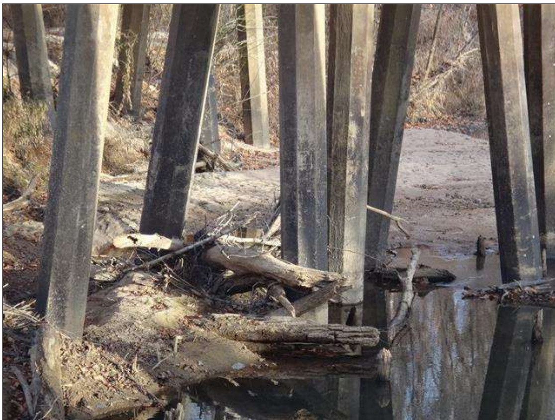
bent 3, drift accumulation (2cy)
