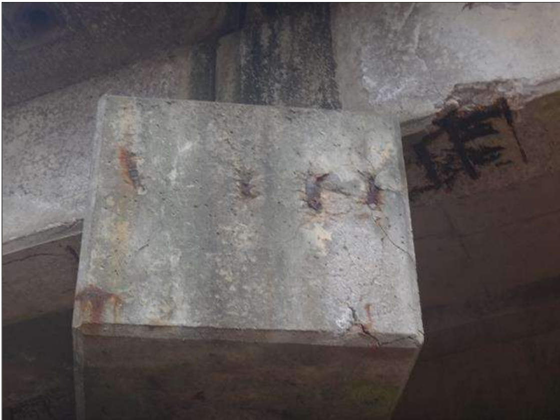
Bent 6 Cap 1: at west face of cap, several spalls with exposed rebar with no measurable section loss (4" high x 2" wide x 1/2" deep.)
