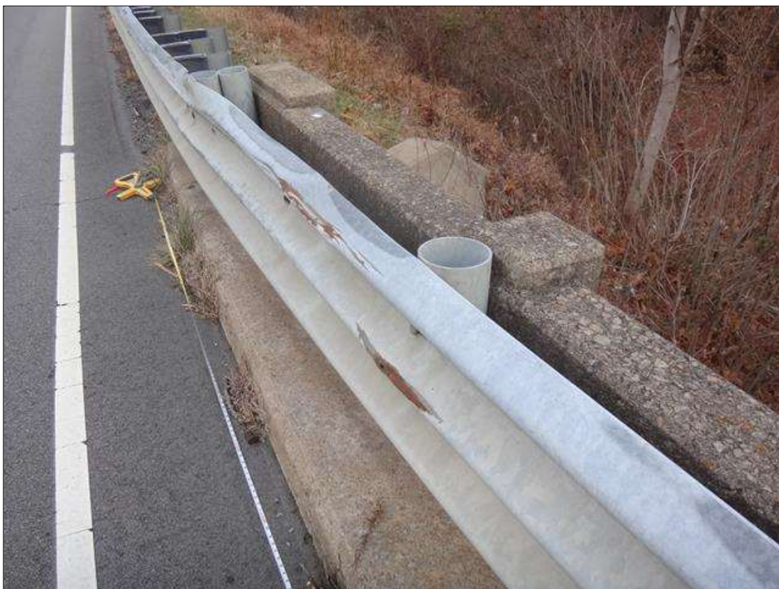
northeast guardrail at end bent 2, impact damage (10ft)
