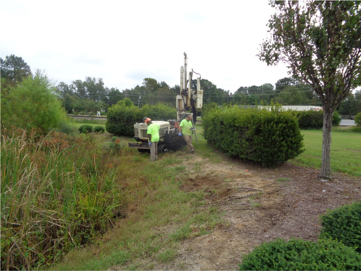
Photo 4 – A view of the southeastern portion of the former canopy/dispenser island area. Stormwater control device now in this area.
