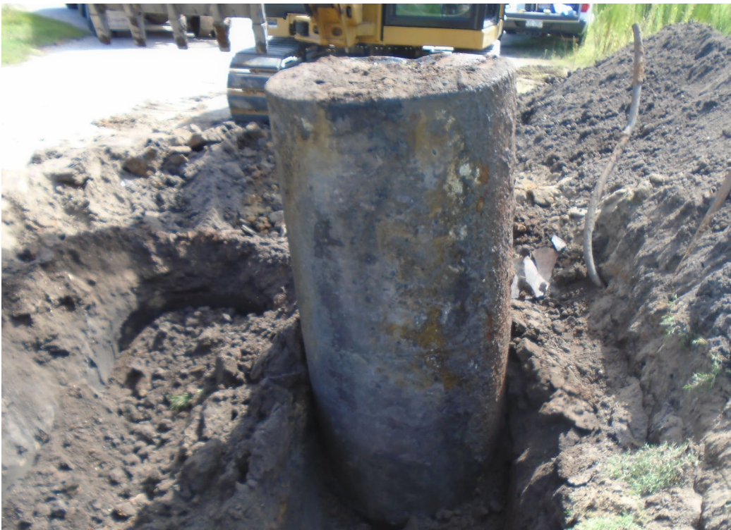
Photograph 6 – Removing the 2 nd 1,000-gallon capacity UST to be hauled off for disposal.
