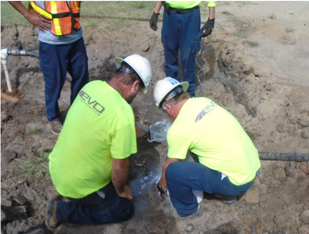
Photograph 4 – Dry ice being added to the USTs prior to checking the LEL and oxygen levels.
