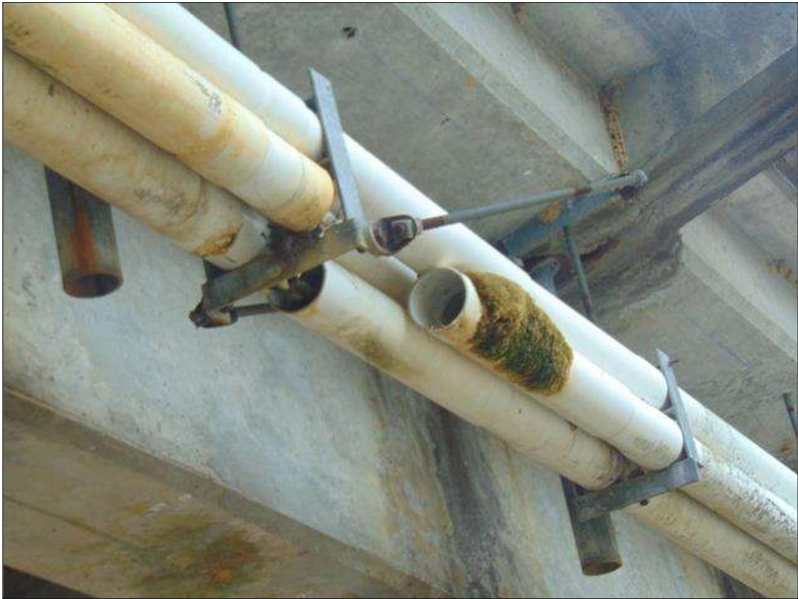
Disconnected utility in Span 5 (Span 4 similar)
