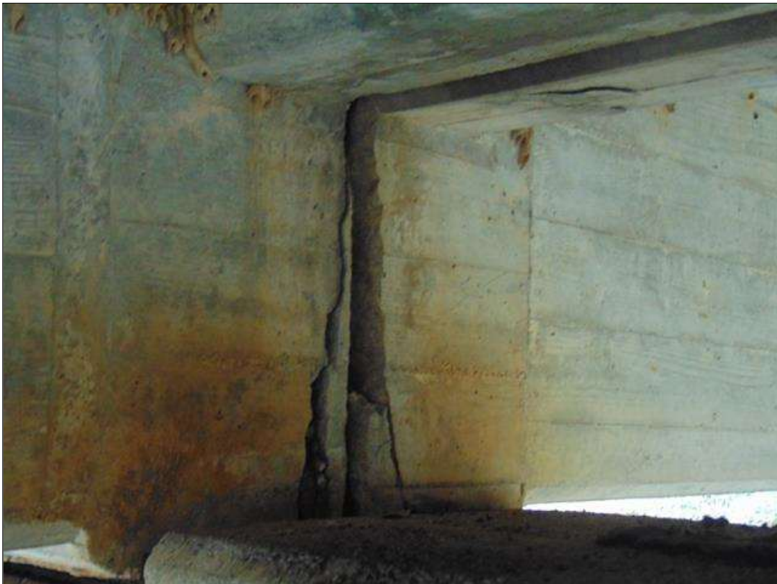
Span 7 Beam 2: 4" LONG x 19" TALL x 3 1/2" DEEP SPALL WITH EXPOSED REBAR ON RIGHT SIDE OF BEAM END AT BENT 6 (PAR)
