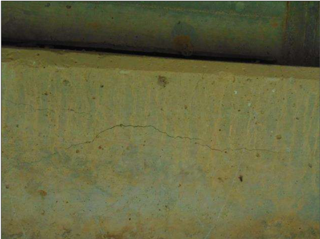
End Bent 2 Cap 1: 2.5' x 8" x 5" DELAMINATION AND 1/16" CRACKING IN Bay 1
