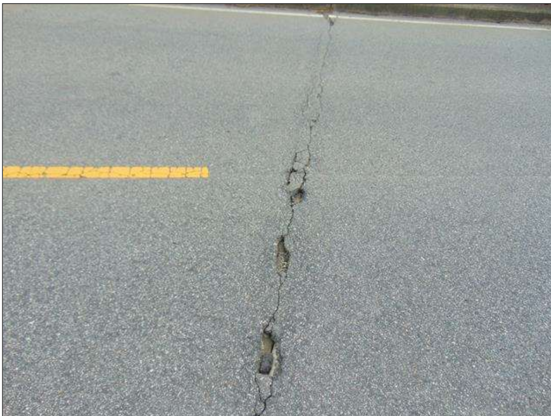
Span 7 Wearing Surface: 30 square feet up to 1/8" transverse crack with (4) up to 12" x 3" x 2" deep area of missing asphalt wearing surface at Bent 6
