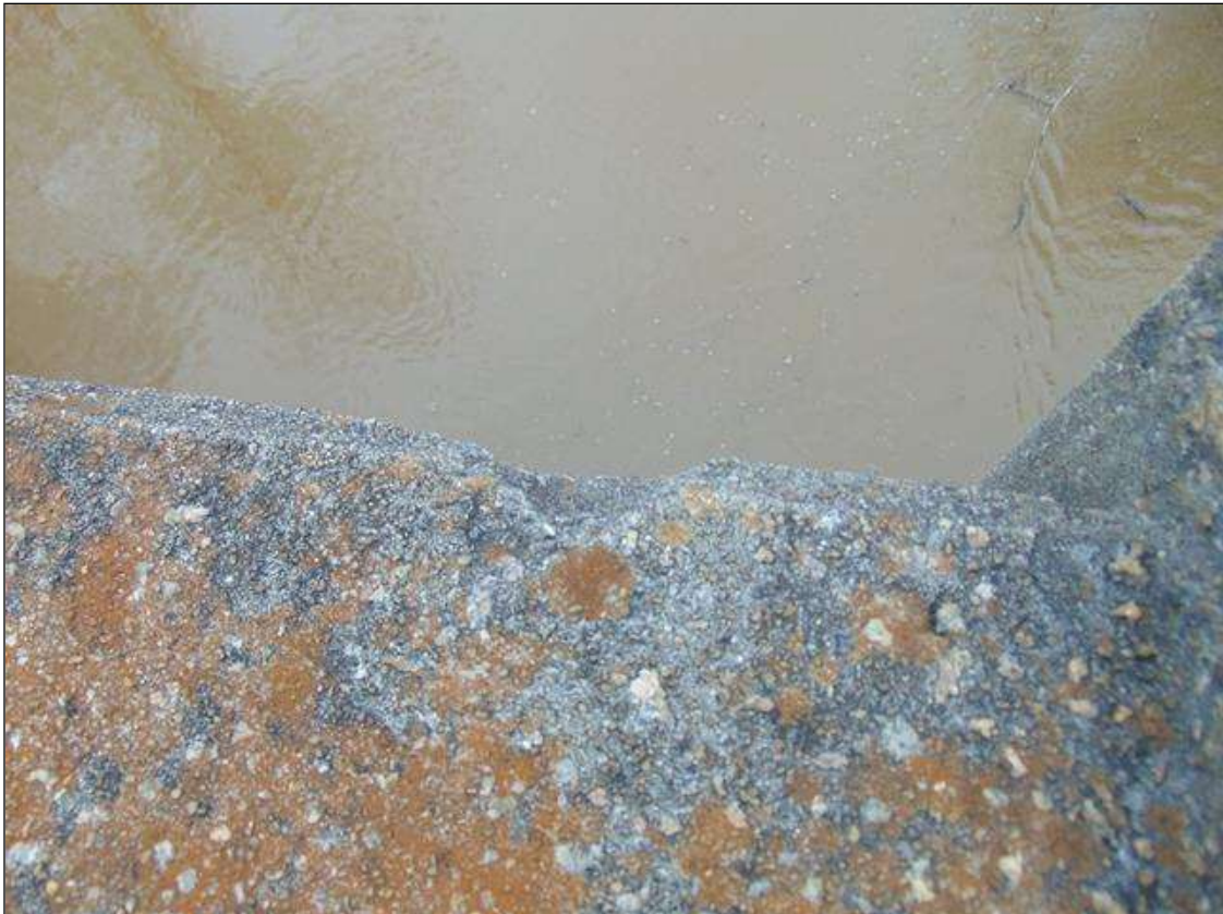
Span 5 Left Bridge Rail: 5" x 4" x 1" deep spall on rail near Post 1
