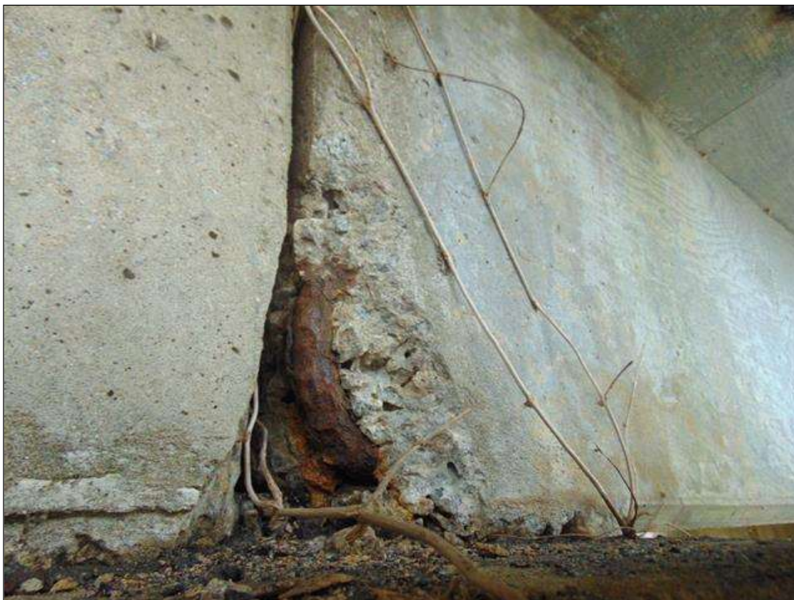
Span 6 Beam 1: [PROMPT ACTION REQUEST] 7" LONG x 12" TALL x 3" DEEP SPALL WITH EXPOSED REBAR ON LEFT SIDE OF BEAM END AT BENT 6, NO MEASURABLE SECTION LOSS
