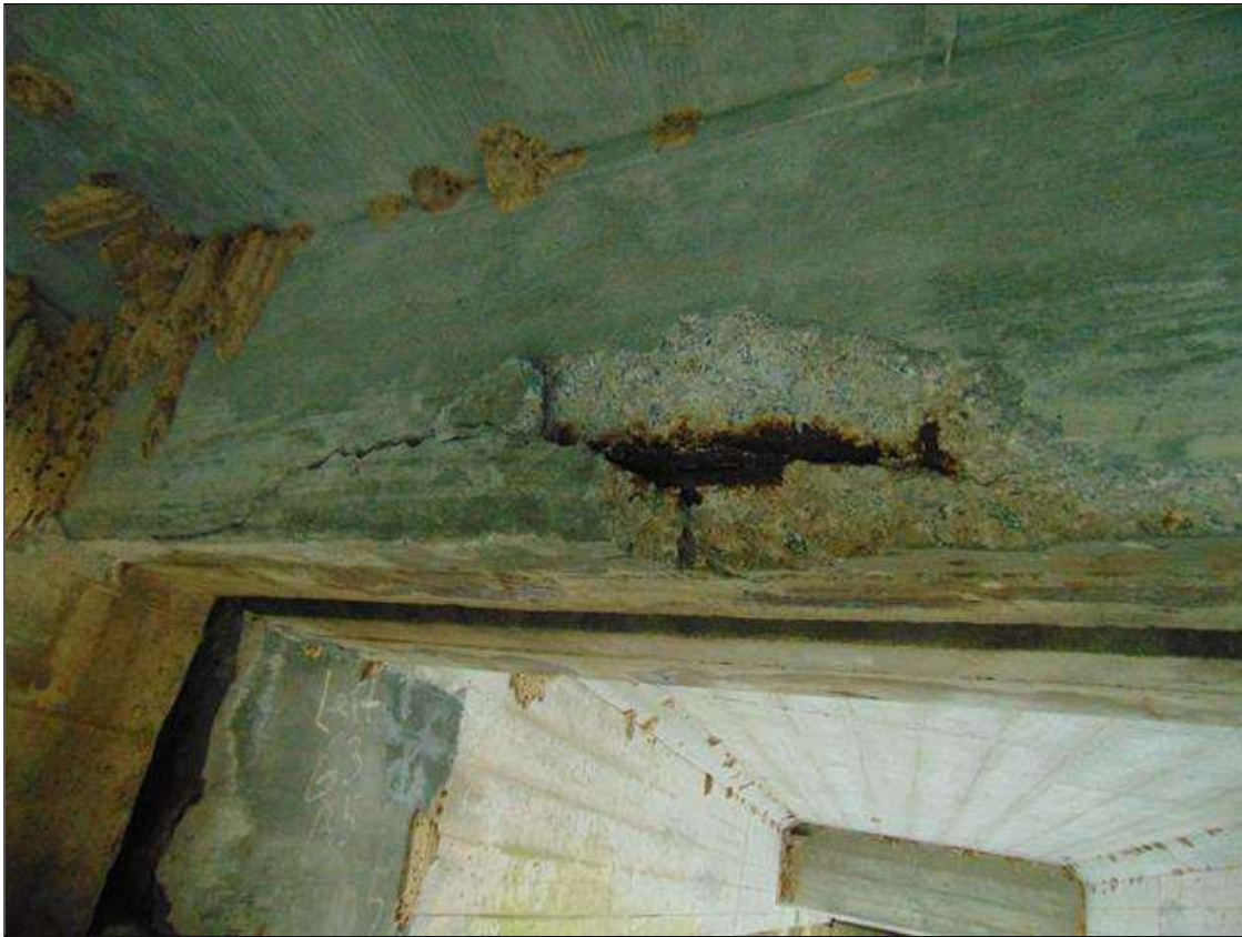
Span 6 Beam 2: 36" x 5" x 2" deep spall with exposed rebar and area of delamination on Bent 5 diaphragm in Bay 2
