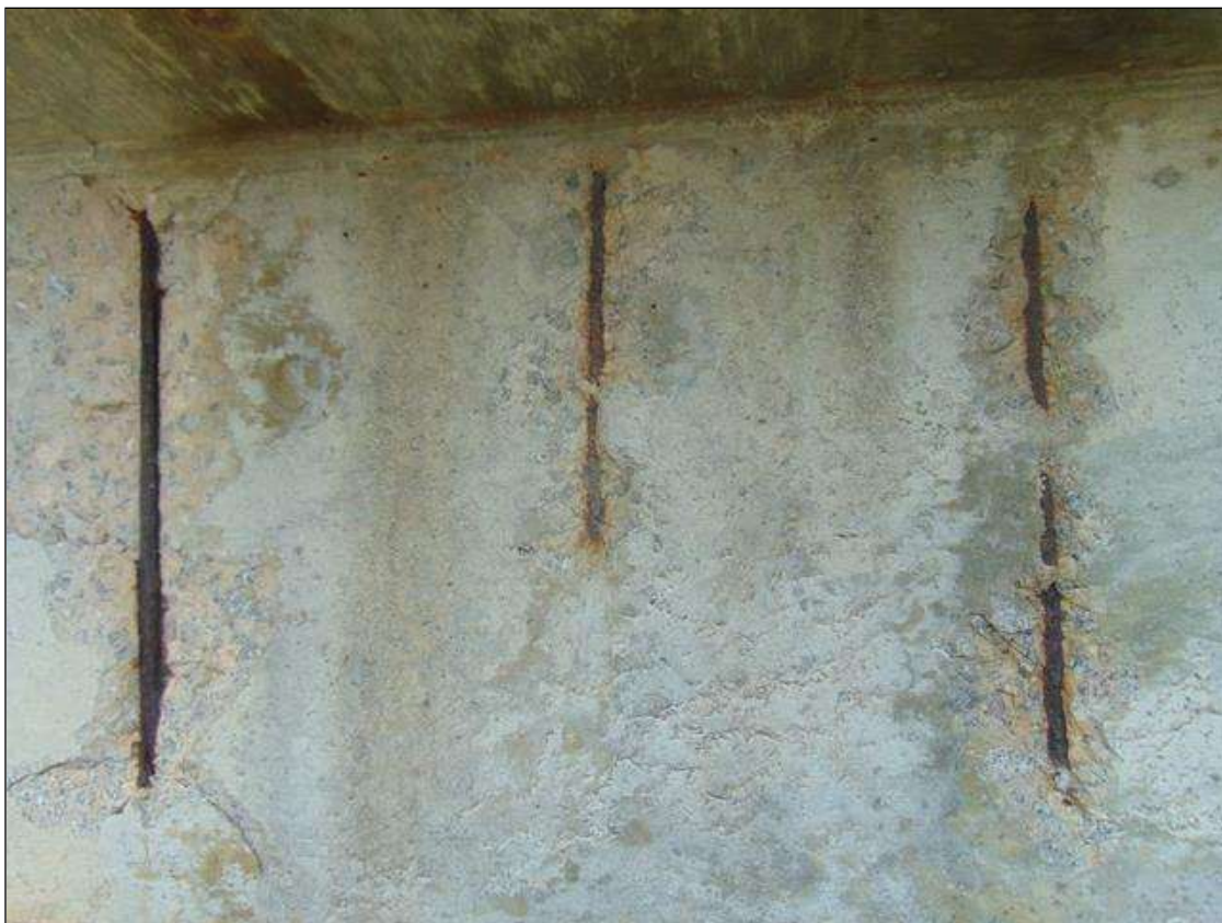
Span 7 Beam 4: 3.5' x 24" x 3/4" DEEP SPALL WITH EXPOSED REBAR ON RIGHT SIDE AT 6' FROM END BENT 2, NO MEASURABLE SECTION LOSS
