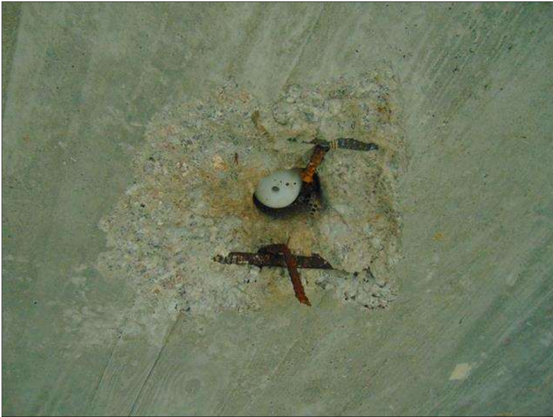
Span 6 Deck: 16" x 14" x 3" deep spall with exposed rebar on bottom of deck in Bay 3 near midspan (Bay 1 similar)
