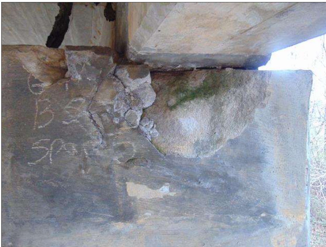
Bent 5 Cap 1: 32" x 14" x 3" DEEP SPALL AND DELAMINATED AREA ON WEST FACE UNDER GIRDER 4 (PAR)
