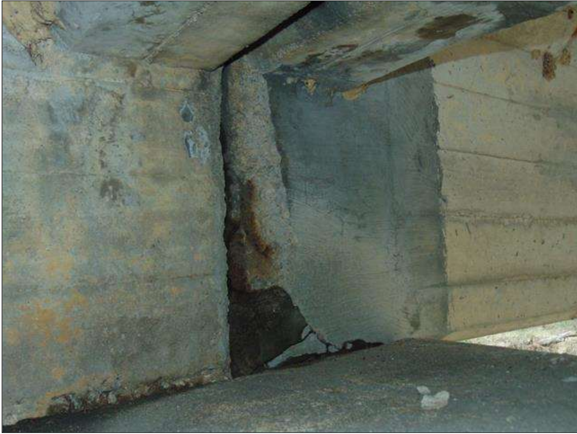
Span 4 Beam 2: [PROMPT ACTION REQUEST] 8" x 18" x 4 1/2" DEEP SPALL WITH EXPOSED REBAR WITH 19" x 19" AREA OF PATCH ON LEFT SIDE OF BEAM END AT BENT 4; RIGHT SIDE SIMILAR
