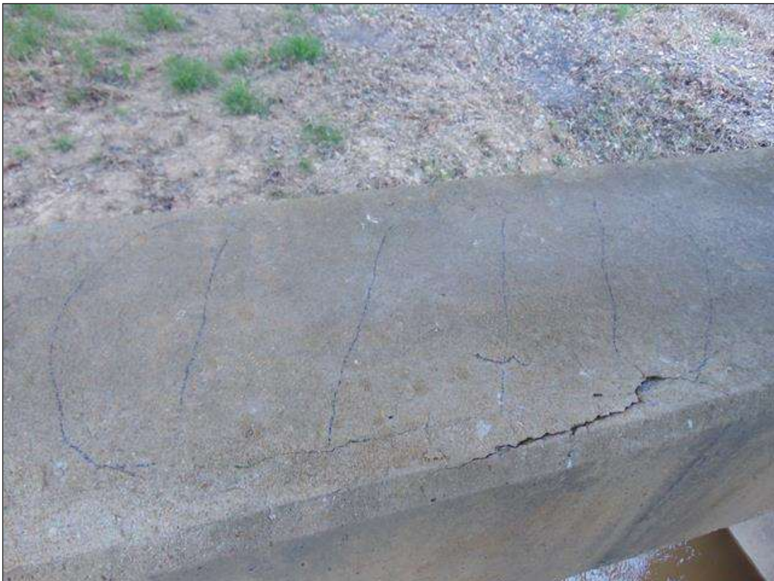
Bent 2 Pile 2: 38" x 18" area of delamination with 1/16" transverse cracks on top of strut between Columns 1 and 2
