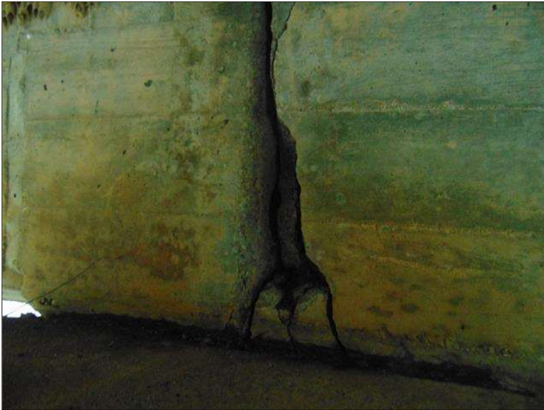
Span 6 Beam 2: [PROMPT ACTION REQUEST] 5" LONG x 19" TALL x 2 1/2" DEEP SPALL WITH EXPOSED REBAR ON BOTH SIDES OF BEAM END AT BENT 6, NO MEASURABLE SECTION LOSS
