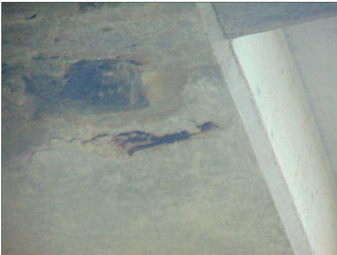
Span 7 Deck: 14" x 9" x 1" DEEP, 8" DIAMETER x 1 1/2" DEEP, AND 2" x 6" x 1/2" DEEP SPALLS ALL EXPOSING REBAR AND AREA OF DELAMINATION IN RIGHT OVERHANG AT DRAIN 4
