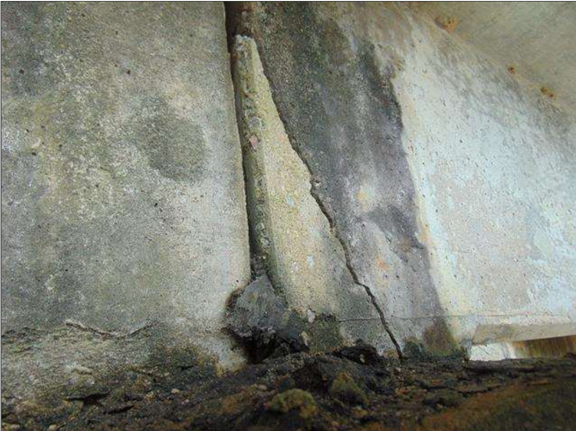
Span 4 Beam 1: GIRDER END AT BENT 4, LEFT SIDE, DIAGONAL CRACKING TO 3/16" WIDE x APPROXIMATELY 15" LONG WITH ASSOCIATED DELAMINATION
