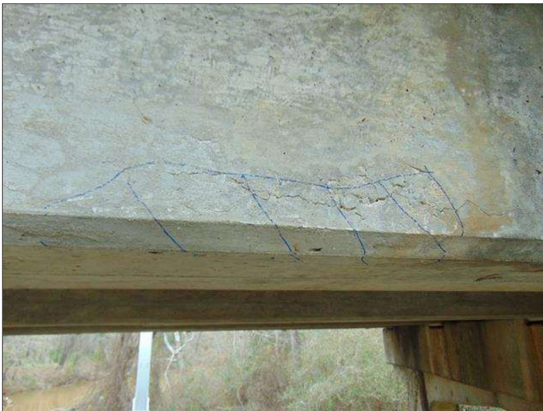
Span 6 Beam 4: 4' x 6" DELAMINATED AREA WITH 1/8" HORIZONTAL CRACKING
