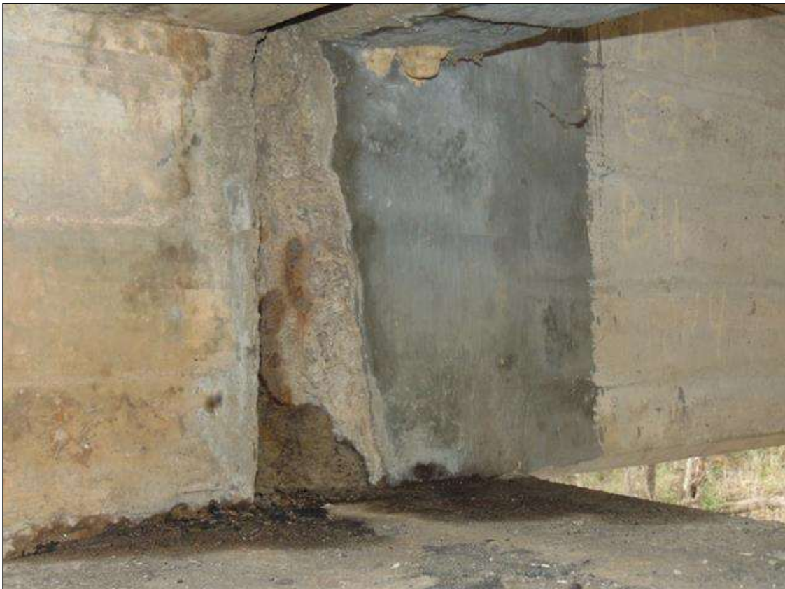
Span 4 Beam 3: [PROMPT ACTION REQUEST] 7" x 9" x 5" DEEP SPALL WITH EXPOSED REBAR WITH 19" x 19" AREA OF PATCH ON LEFT SIDE OF BEAM END AT BENT 4; RIGHT SIDE SIMILAR
