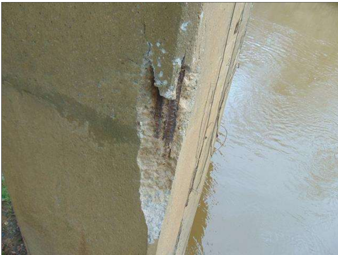
Bent 5 Pile 1: 37" x 5" x 2 1/2" deep spall with exposed rebar and area of delamination on Northeast corner (PAR)
