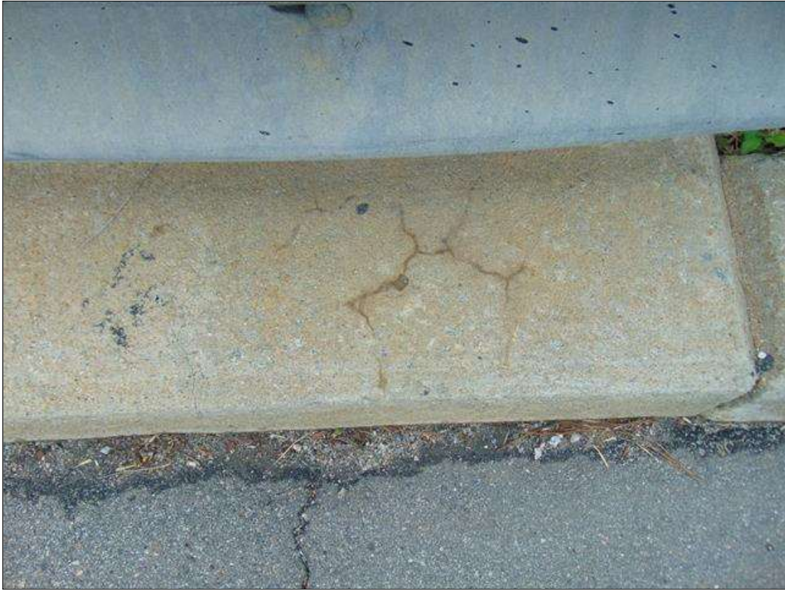
Span 7 Left Bridge Rail: 18" x 12" area of hairline map cracking on curb at End Bent 2
