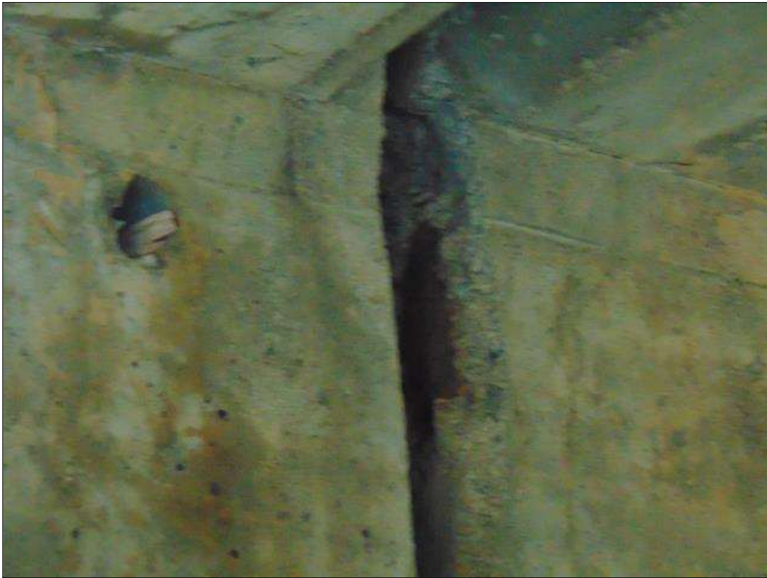
Span 2 Beam 4: 2 1/2" x 5" x 1/2" deep spall with exposed rebar on left side of beam at Bent 2 (PAR)
