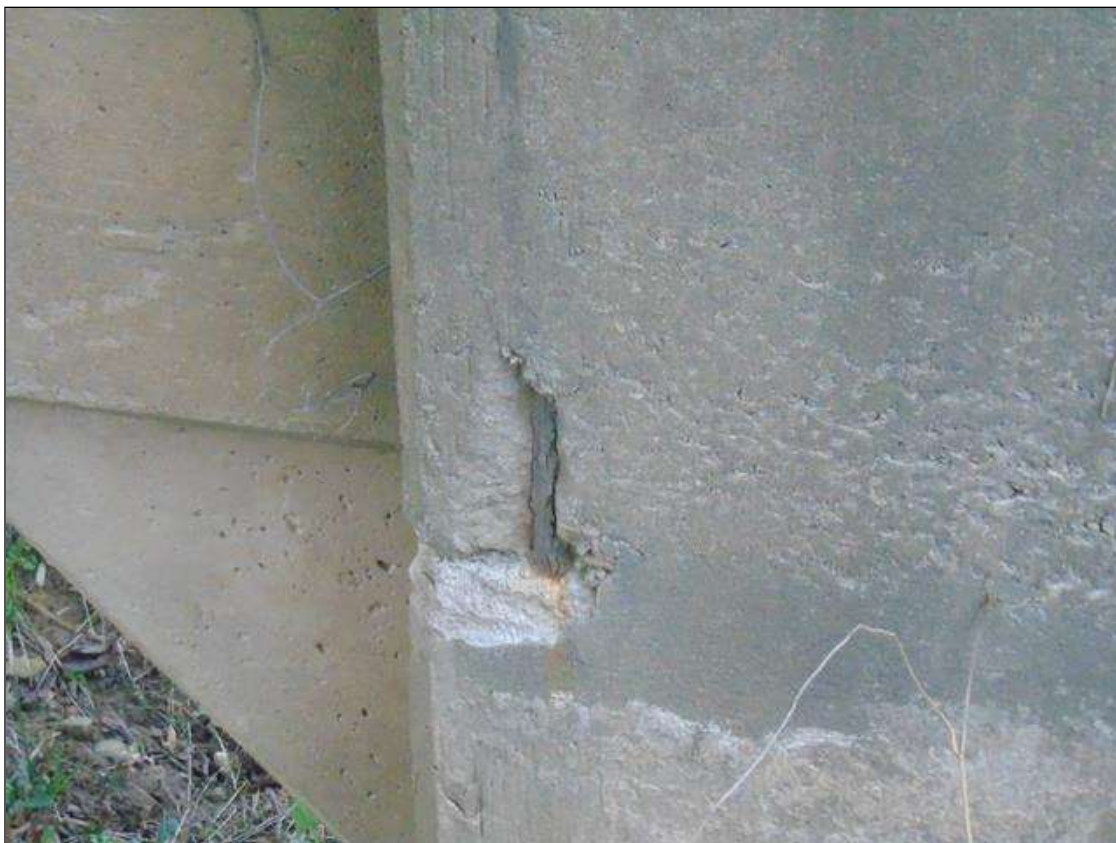
Bent 6 Pile 2: 12" x 6" x 1 1/2" DEEP SPALL WITH EXPOSED REBAR AND AREA OF DELAMINATION ON Northwest CORNER AT STRUT (PAR)
