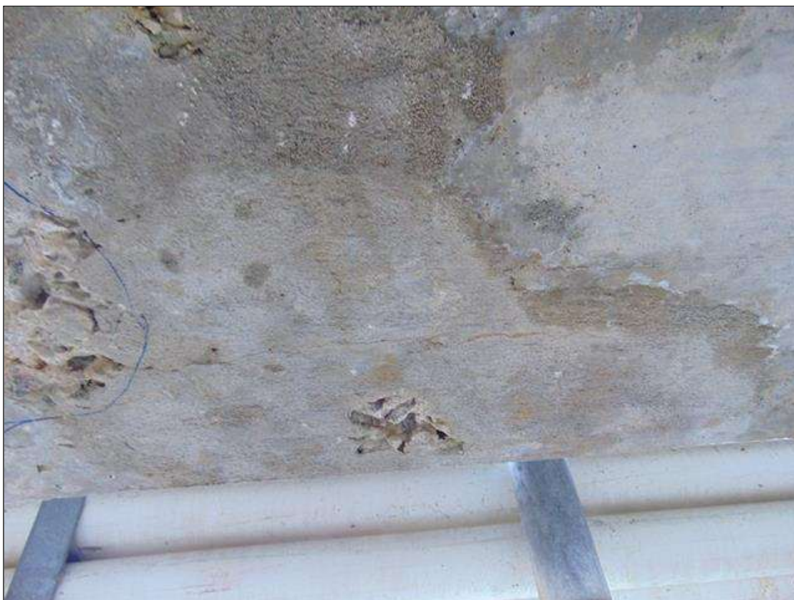
Span 6 Beam 1: 20" x 16" area of patch with 3 1/2" x 3" x 1/2" deep spall on bottom of beam near midspan
