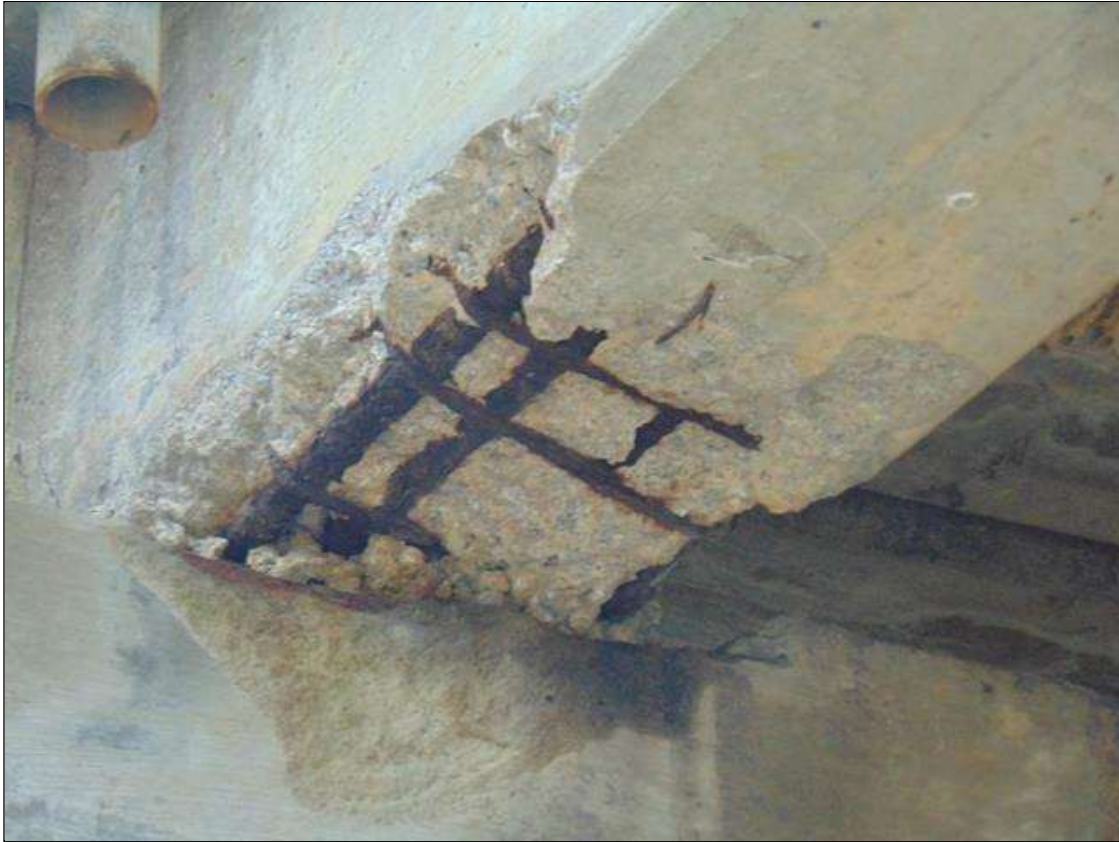
Span 5 Beam 1: [PROMPT ACTION REQUEST] 32" x 18" x 3" DEEP SPALL WITH EXPOSED REBAR ON BOTTOM OF GIRDER WITH 12" x 4" x 5" DEEP SPALL ON LEFT SIDE OF BEAM END AT BENT 5 WITH VOIDS RESULTING FROM POOR CONSOLIDATION. APPROXIMATELY 50% OF BEARING AREA HAS BEEN LOST. THERE IS UP TO 50% SECTION LOSS ON THE SECONDARY REINFORCING.
