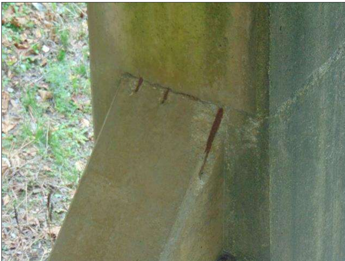
Bent 1 Pile 1: EAST FACE ON THE STRUCT, SPALLING WITH EXPOSED REBAR [APPROXIMATELY (3) UP TO 12" x 4" x 1" DEEP], NO MEASURABLE SECTION LOSS
