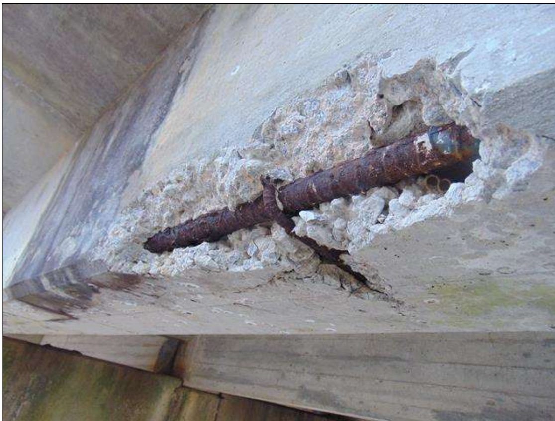
Span 5 Beam 4: [PROMPT ACTION REQUEST] 3' x 15" x 5" DEEP SPALL WITH EXPOSED REBAR ON UNDERSIDE AT 15' FROM BENT 4, NO MEASURABLE SECTION LOSS
