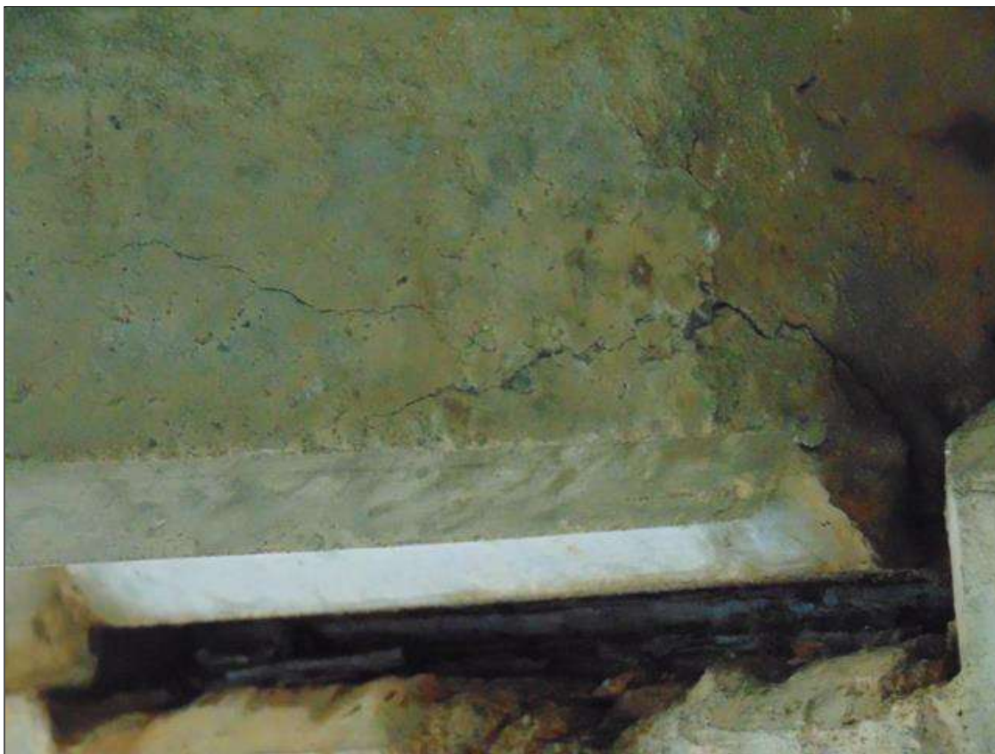
Span 6 Beam 3: (2) up to 11" long 1/16" horizontal cracks on right side of beam at Bent 6
