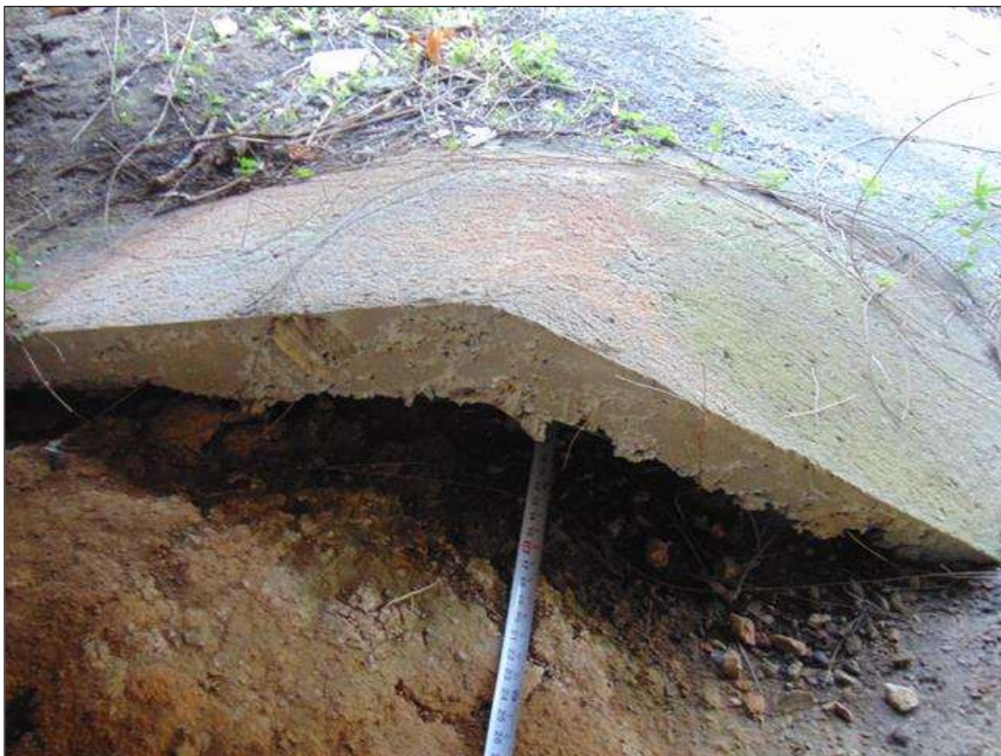
4' x 1' deep undermining under End Bent 1 slope protection at North end (South end similar) (PAR)
