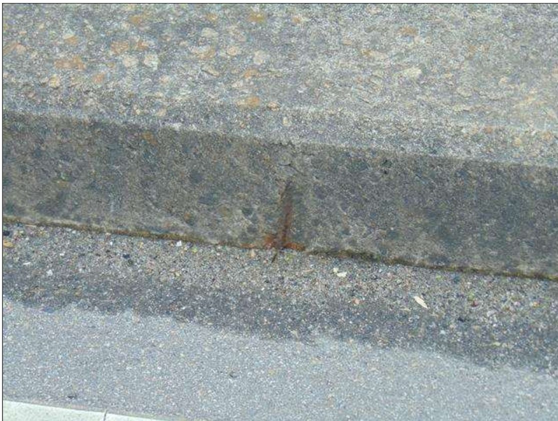
Span 5 Right Bridge Rail: (5) up to 4 1/2" x 2" x 1/2" deep spalls with exposed rebar on curb face
