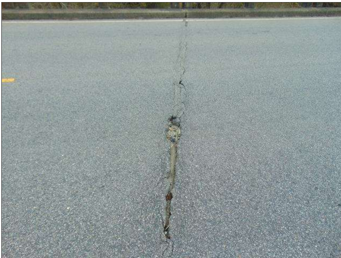
Span 6 Wearing Surface: Full width transverse crack with (2) up to 56" x 6" x 2" deep area of missing asphalt wearing surface at Bent 5
