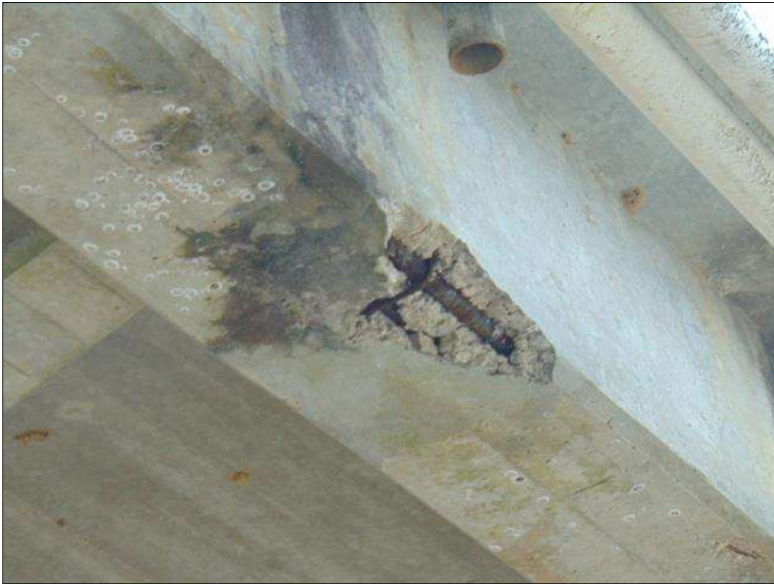
Span 5 Beam 1: [PROMPT ACTION REQUEST] 26" x 14" x 3 1/2" DEEP SPALL WITH EXPOSED REBAR ON UNDERSIDE AT MIDSPAN. THERE ARE VOIDS AROUND THE REBAR AS A RESULT OF POOR CONSOLIDATION. THE SECONDARY REINFORCING HAS UP TO 50% SECTION LOSS.
