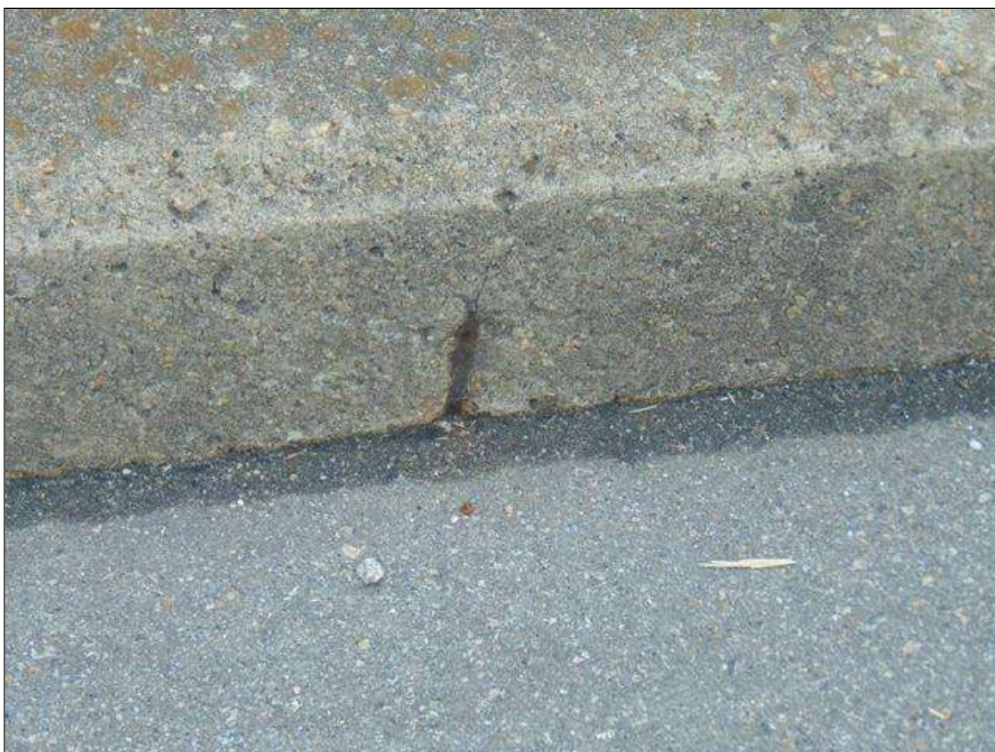
Span 1 Left Bridge Rail: (3) UP TO 5" x 1" x 1/4" DEEP SPALLS WITH EXPOSED REBAR ON CURB NEAR POST 7
