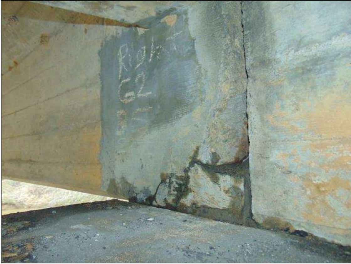
Span 5 Beam 2: [PROMPT ACTION REQUEST] 6" LONG x 18" TALL x 4" DEEP SPALL WITH EXPOSED REBAR WITH ADJACENT 16" x 10" AREA OF PATCH ON RIGHT SIDE OF BEAM END AT BENT 5, NO MEASURABLE SECTION LOSS
