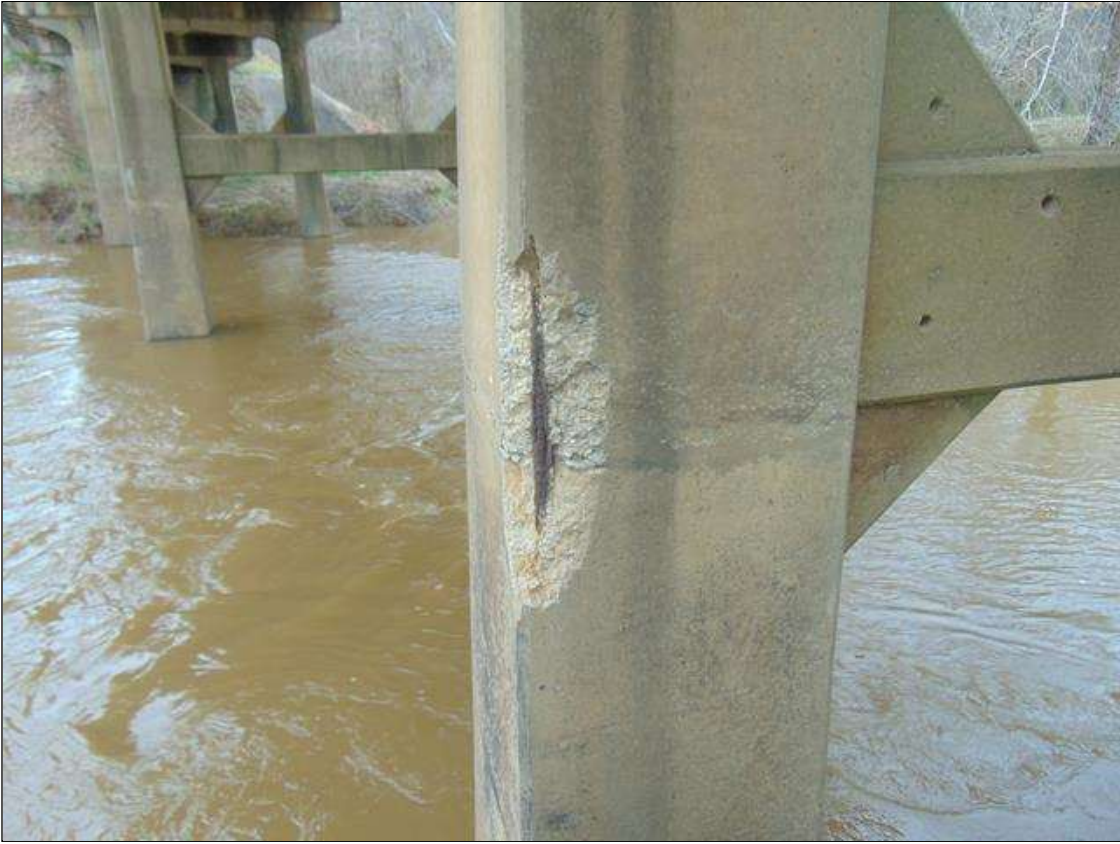
Bent 4 Pile 2: [PROMPT ACTION REQUEST] 4.5' x 7" x 8" DEEP SPALL WITH EXPOSED REBAR ON Southeast CORNER
