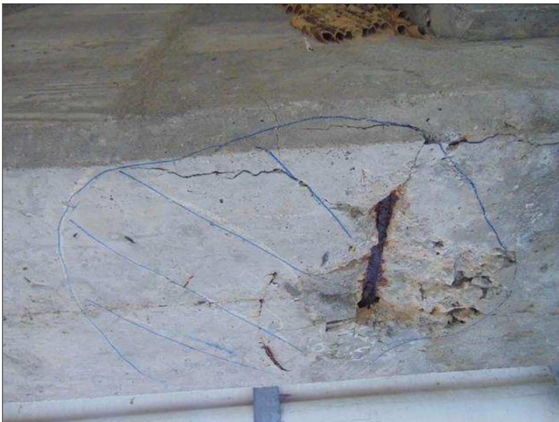
Span 6 Beam 1: 16" x 14" x 1" deep spall with exposed rebar and area of delamination on bottom of beam near midspan
