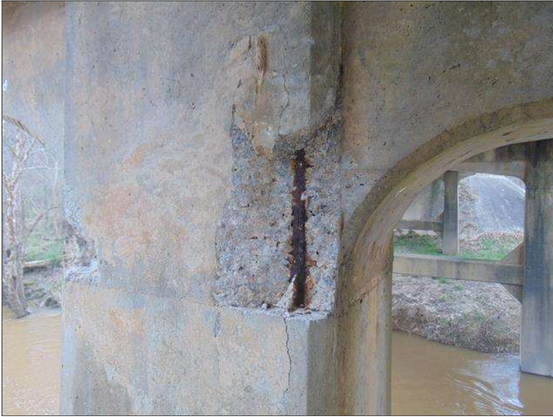
Bent 3 Pile 2: [PROMPT ACTION REQUEST] 2' DOWN FROM CAP, [2] AREAS OF SPALLING WITH EXPOSED REBAR AND AREA OF DELAMINATION UP TO 3' HIGH x 12" WIDE x 3" DEEP WITH NO MEASURABLE SECTION LOSS ON Span 4 FACE
