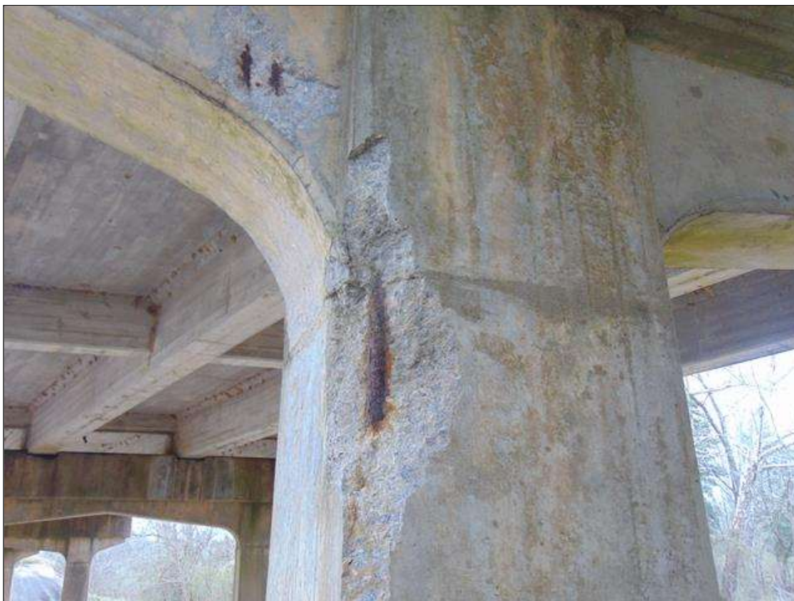
Bent 2 Pile 1: 44" x 9" x 8" SPALL WITH EXPOSED REBAR ON Northwest CORNER (PAR)
