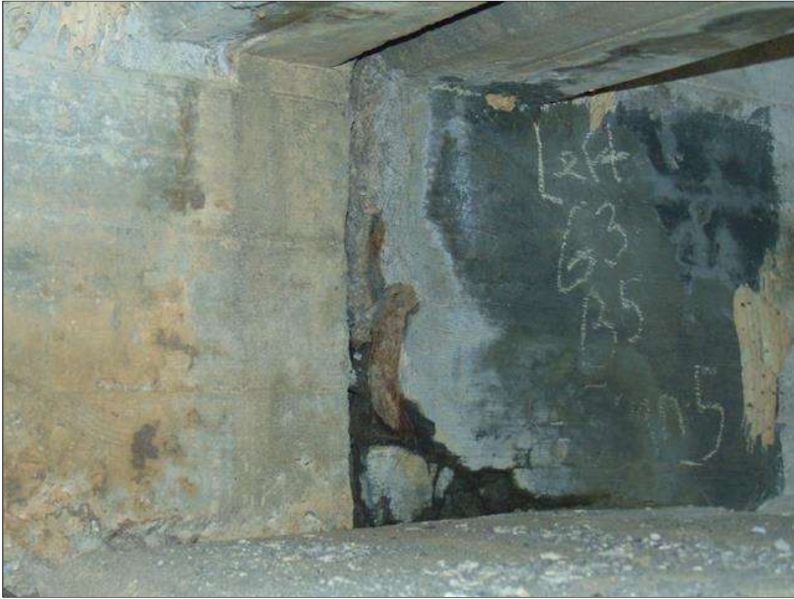
Span 5 Beam 3: [PROMPT ACTION REQUEST] 7" LONG x 18" TALL x 5" DEEP SPALL WITH EXPOSED REBAR WITH ADJACENT 16" x 20" AREA OF PATCH ON LEFT SIDE OF BEAM END AT BENT 5, NO MEASURABLE SECTION LOSS
