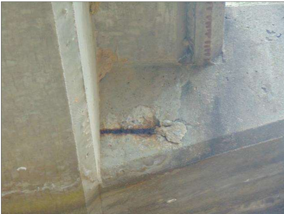
Span 5 Right Bridge Rail: 8" x 3" x 1/2" deep spall with exposed rebar on West face of Post 6 bracket
