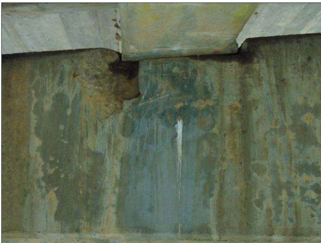
Bent 2 Cap 1: 20" x 12" x 8" DEEP SPALL AND DELAMINATED AREA ON WEST FACE UNDER GIRDER 3
