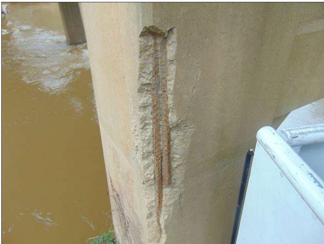
Bent 5 Pile 2: [PROMPT ACTION REQUEST] 4.75' x 8" x 8" SPALL WITH EXPOSED REBAR AND AREA OF DELAMINATION ON Southeast CORNER
