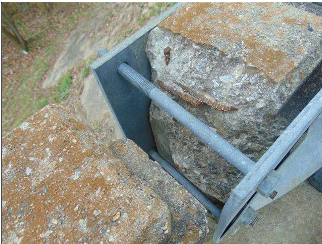
Span 1 Right Bridge Rail: 12" x 11" x 5" DEEP SPALL WITH EXPOSED REBAR ON POST 2
