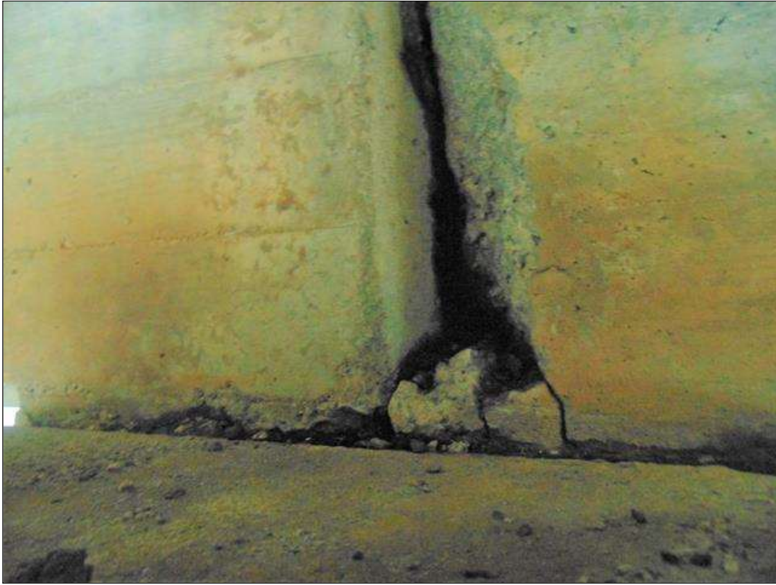
Span 6 Beam 3: [PROMPT ACTION REQUEST] 5" LONG x 19" TALL x 4" DEEP SPALL WITH EXPOSED REBAR [NO MEASURABLE SECTION LOSS] ON LEFT SIDE OF BEAM END AT BENT 6 AND 8" LONG x 10" TALL x 2 1/2" DEEP SPALL WITH EXPOSED REBAR [NO MEASURABLE SECTION LOSS] ON RIGHT SIDE OF BEAM END OVER BENT 6
