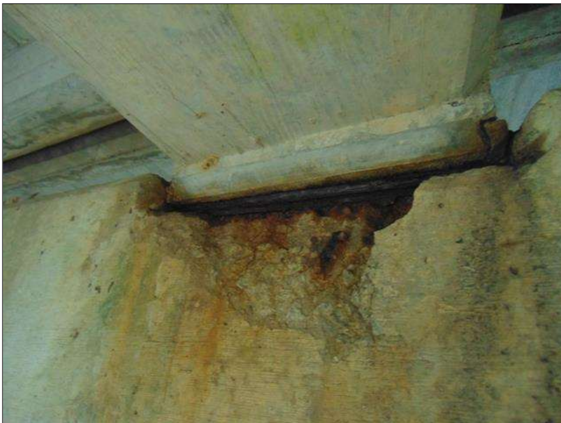
Bent 6 Cap 1: 18" x 9" x 3" DEEP SPALL WITH EXPOSED REBAR ON EAST FACE UNDER GIRDER 3 (PAR)
