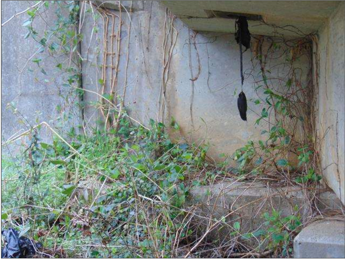
Vegetation growth on End Bent 1 cap at South end
