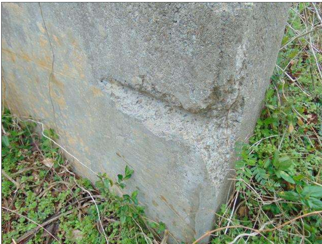
14" x 13" x 1 1/2" deep spall on Southeast wingwall
