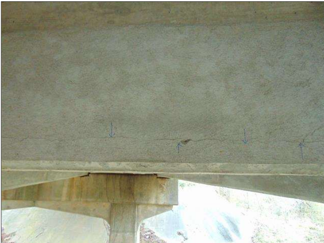
Span 6 Beam 3: 4' hairline horizontal crack on West face of intermediate diaphragm in Bay 3
