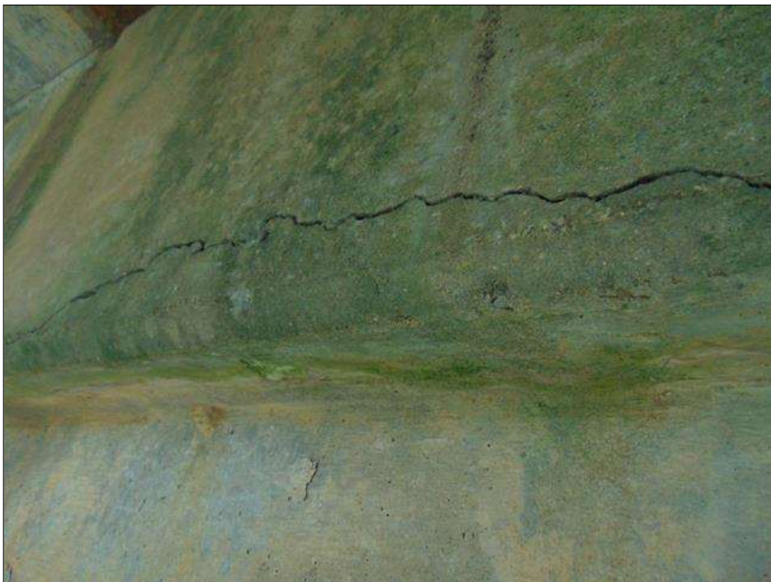
Bent 5 Cap 1: 40" x 7" AREA OF DELAMINATION WITH 1/8" HORIZONTAL CRACK ON EAST FACE UNDER Bay 2
