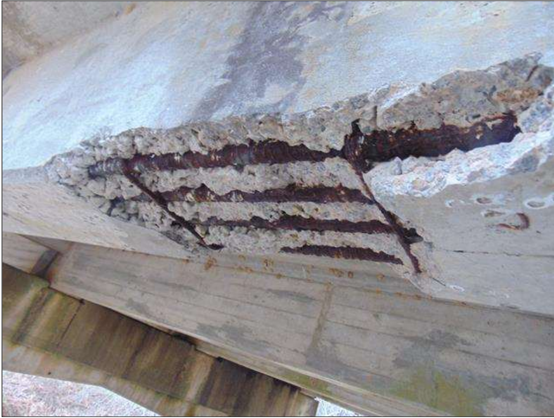
Span 5 Beam 4: [PROMPT ACTION REQUEST] 3.5' x 18" x 4" DEEP SPALL WITH EXPOSED REBAR ON UNDERSIDE AT MIDSPAN. THERE ARE VOIDS IN THE CONCRETE RESULTING FROM POOR CONSOLIDATION. THE SECONDARY REINFORCING HAS UP TO 50% SECTION LOSS.
