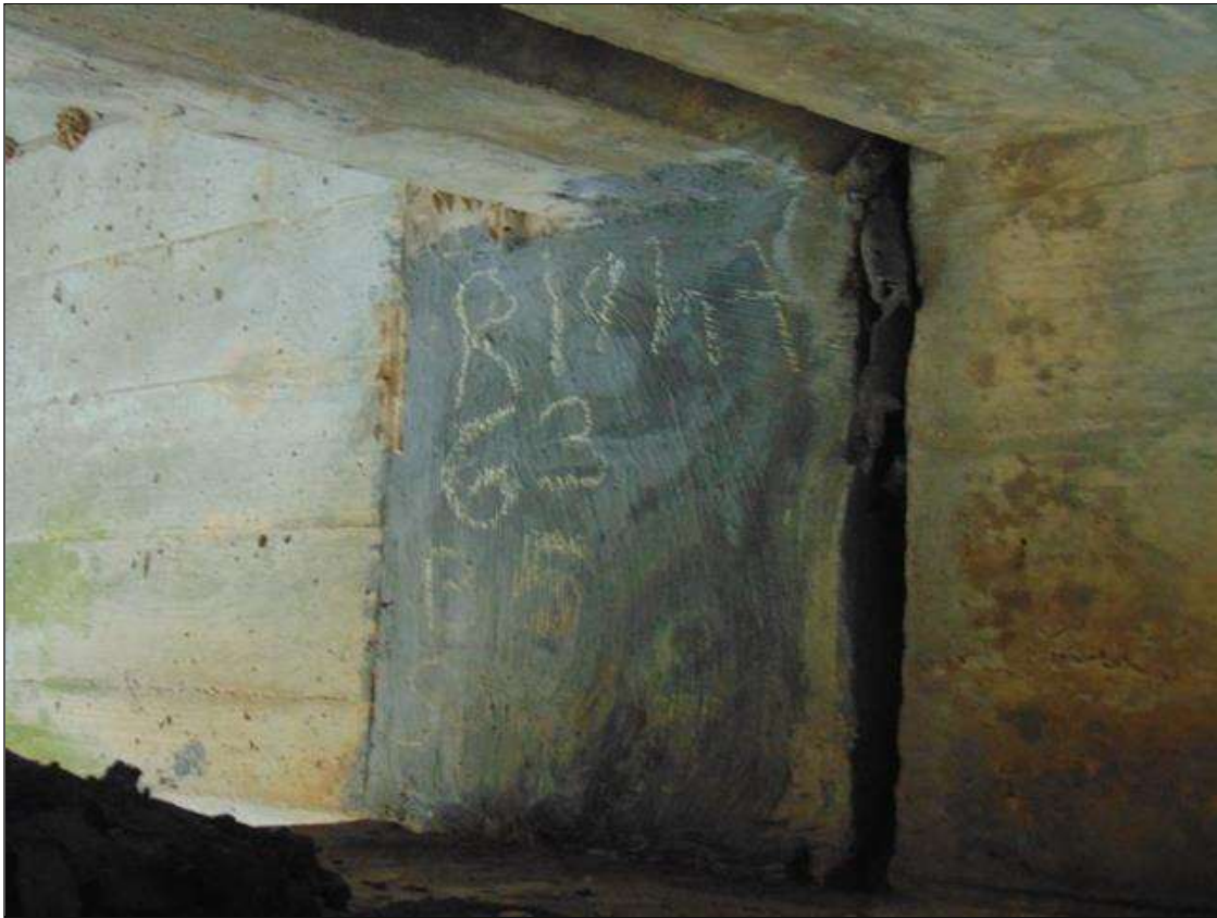
Span 5 Beam 3: 14" x 18" area of sound patch on right side of beam at Bent 5
