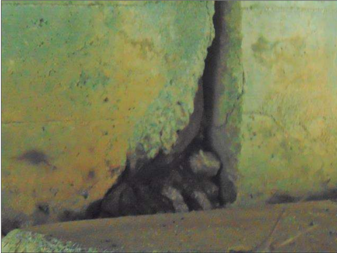
Span 6 Beam 3: [PROMPT ACTION REQUEST] 5" LONG x 19" TALL x 4" DEEP SPALL WITH EXPOSED REBAR [NO MEASURABLE SECTION LOSS] ON LEFT SIDE OF BEAM END AT BENT 6 AND 8" LONG x 10" TALL x 2 1/2" DEEP SPALL WITH EXPOSED REBAR [NO MEASURABLE SECTION LOSS] ON RIGHT SIDE OF BEAM END OVER BENT 6
