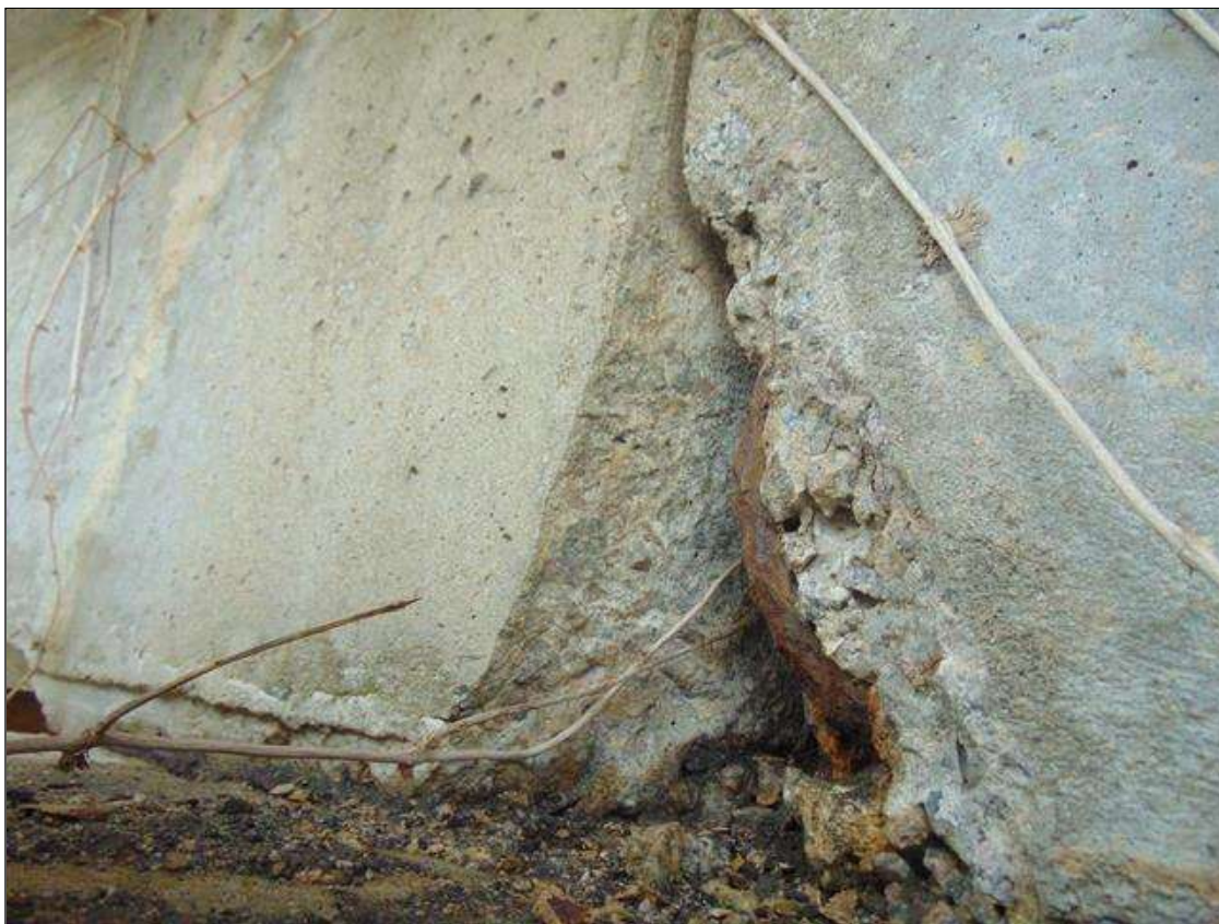
Span 7 Beam 1: 2" x 11" x 4" deep spall with exposed rebar on left side of beam at Bent 6 (PAR)
