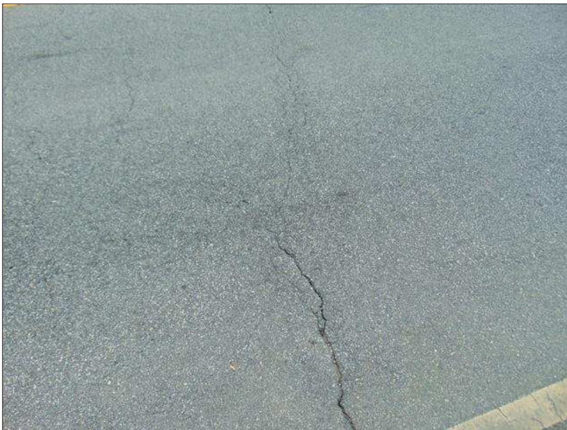
Span 7 Wearing Surface: 30 square feet up to 1/8" transverse crack at End Bent 2
