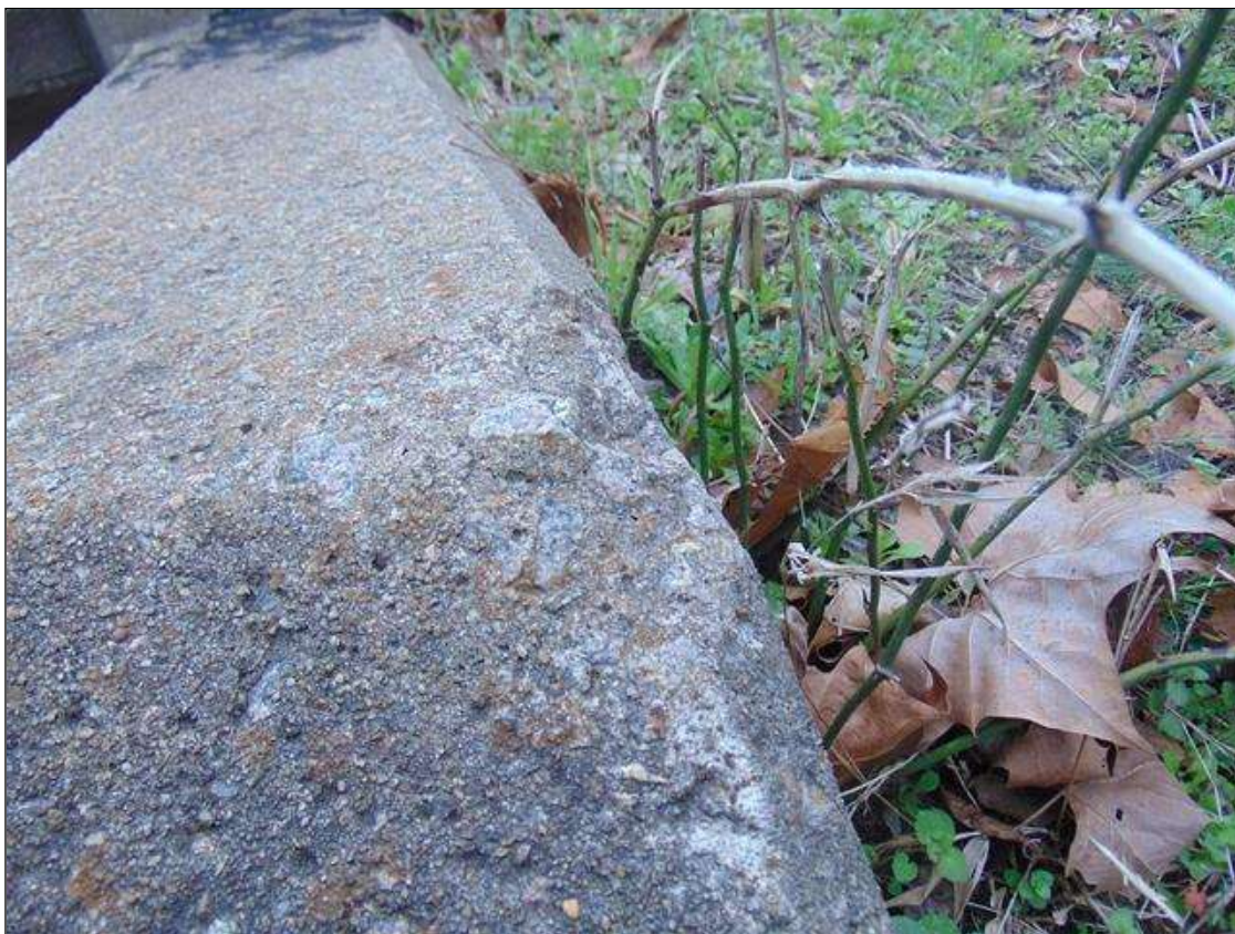
(2) up to 5" x 2" x 1" deep spalls on Northwest wingwall
