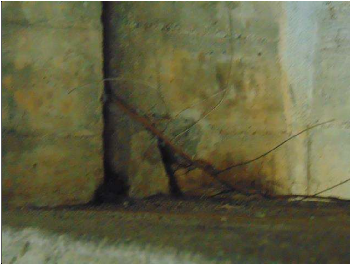
Span 1 Beam 4: 6" LONG x 6" TALL SPALLING UP TO 2" DEEP AND ARE OF DELAMINATION ON BEAM END OVER BENT 1, LEFT SIDE
