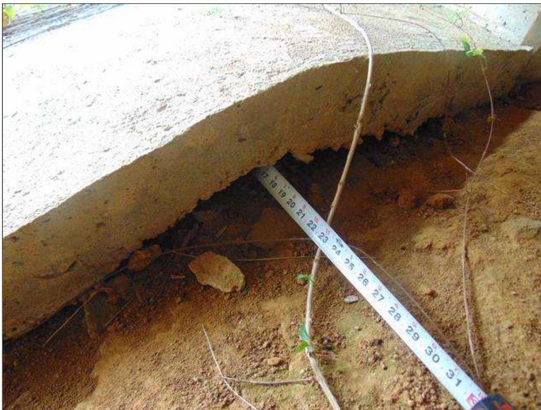
2' x 18" deep undermining under End Bent 2 slope protection at North end (South end similar) (PAR)
