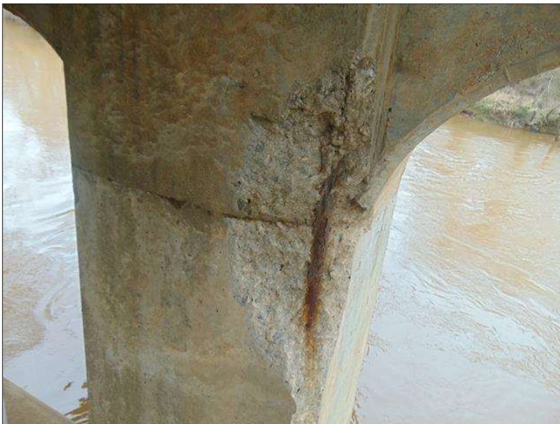
Bent 2 Pile 2: [PROMPT ACTION REQUEST] 50" x 10" x 8" SPALL WITH EXPOSED REBAR ON Southwest CORNER
