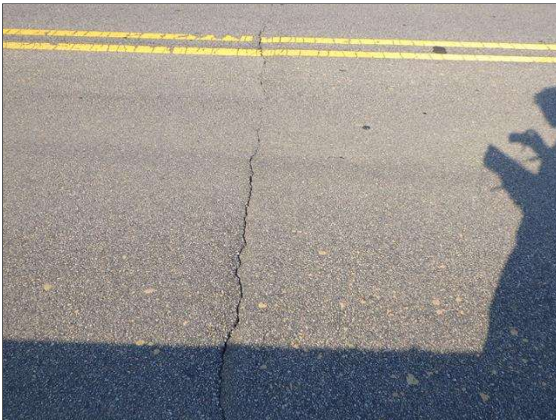
Span 2 Wearing Surface: UP TO 1/8" TRANSVERSE CRACKING OVER BENT 1
