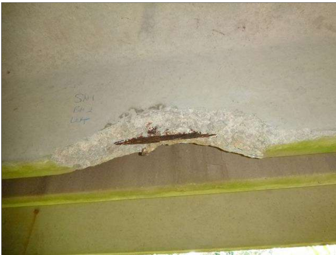
Span 1 Slab 2: [PAR] left leg near midspan, spall [16in x 5in x full width] with exposed strand that exhibits section loss [up to 25%]
