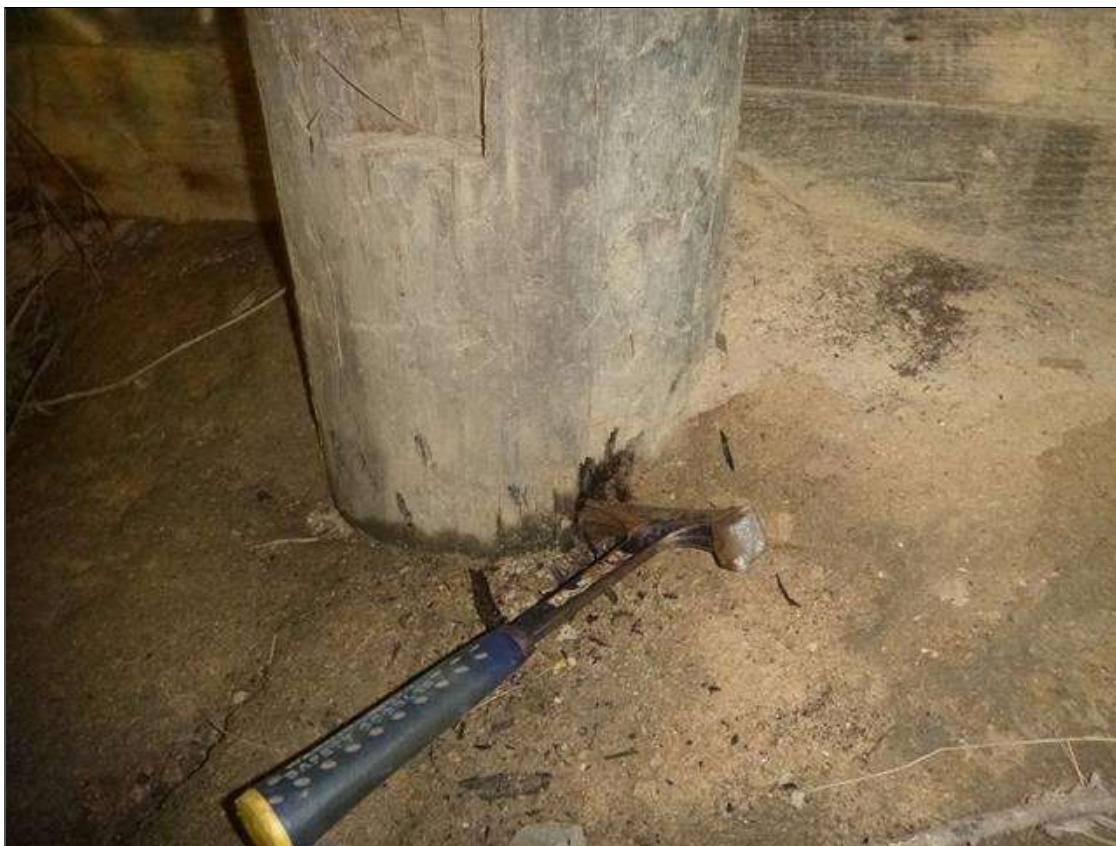
End Bent 2 Pile 3: at base of pile, decay (8in x 1in x 1-1/2in deep)
