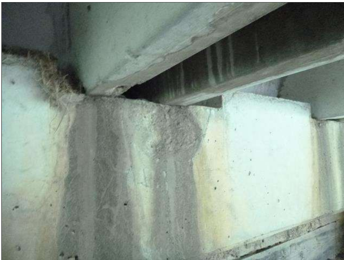
End Bent 1 Cap 1: over pile 3, spall/delamination [8in x 5in x 1/4in deep]
