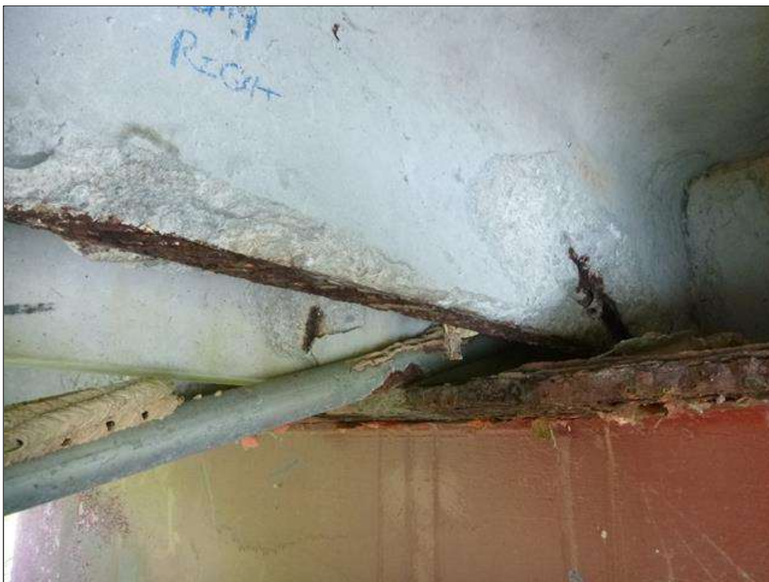
Span 2 Slab 9: [PAR] right leg at bent 1, spall/delamination [52in x 8in x up to full width] with one exposed strand (50% section loss on strand)
