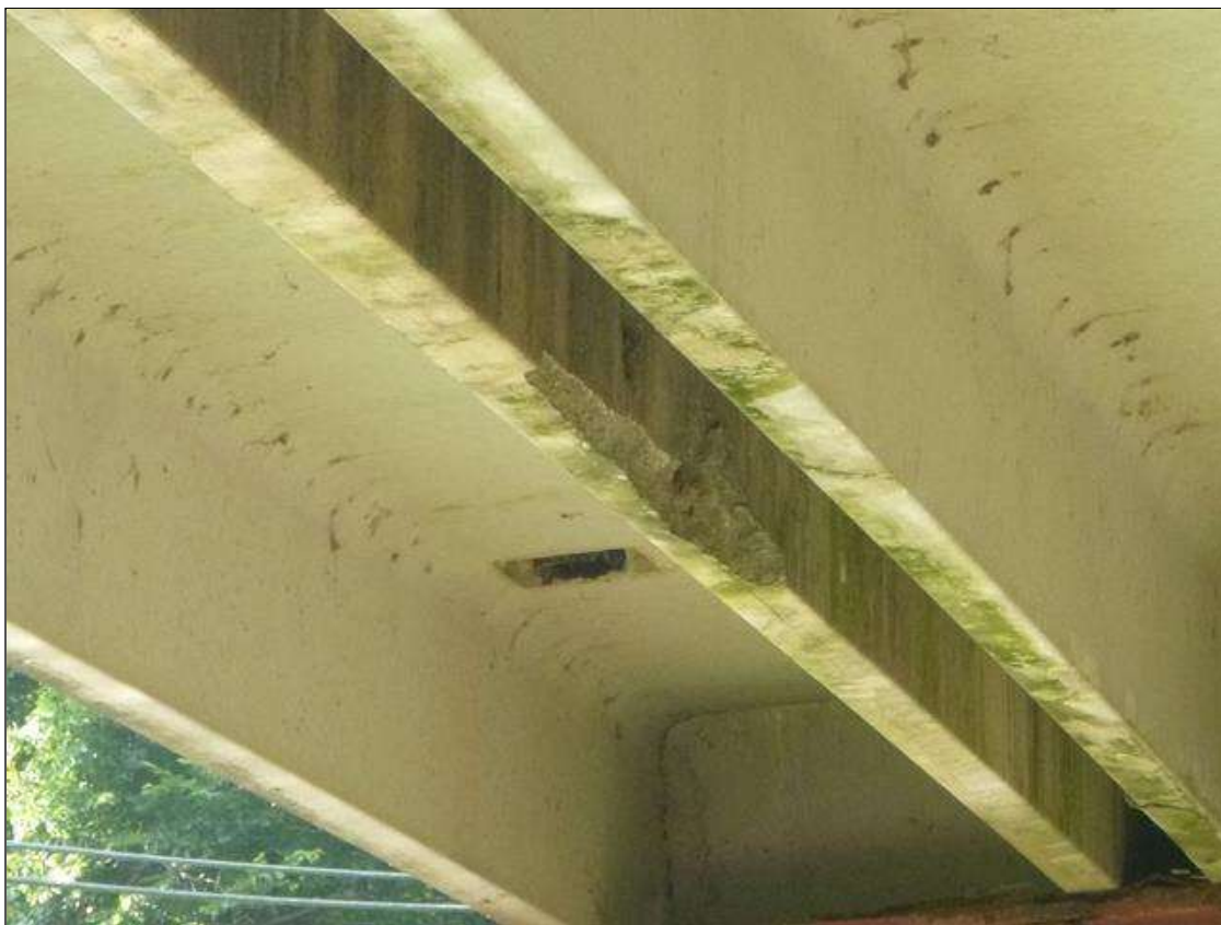
Span 2 Slab 1: right leg 6ft from bent 2, spall (30in x 3in x 3/4in) with exposed rusted rebar
