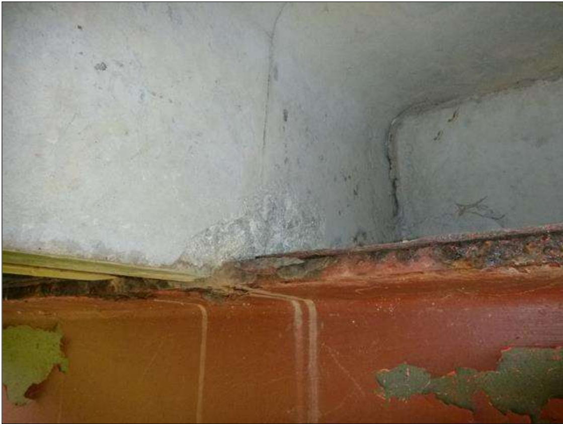
Span 1 Slab 2: (PAR) left and right leg at bent 1, three [3] spalls/delaminations [up to 10in x 6in x 1in deep] channel legs crushing and bottom of channel legs sits below top of crutch bent cap
