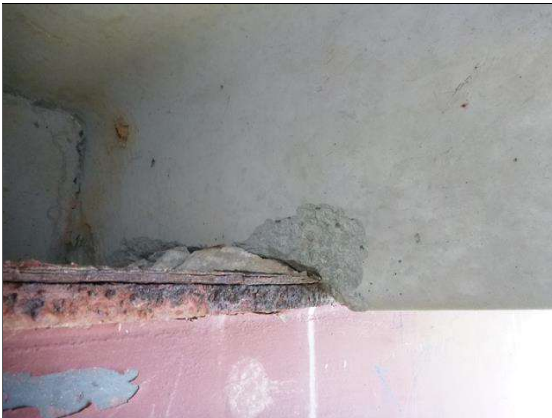
Span 2 Slab 5: (PAR) left and right leg at bent 1, two [2] spalls [up to 12in x 8in x up to full width], with exposed stirrup [no section loss noted] channel legs crushing and bottom of channel legs sits below top of crutch bent cap (photo 1 of 2)
