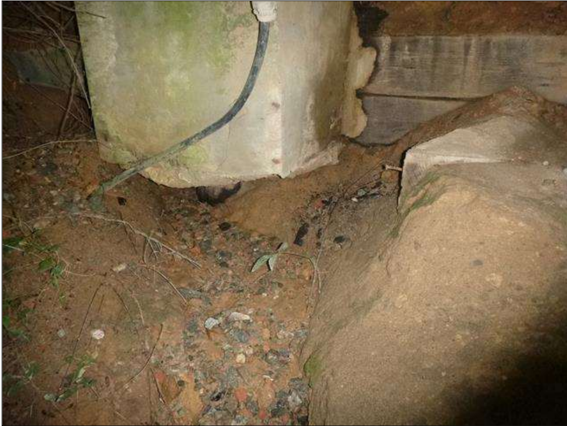
End Bent 1 Pile 5: (PAR) concrete collar is undermined (60%)
