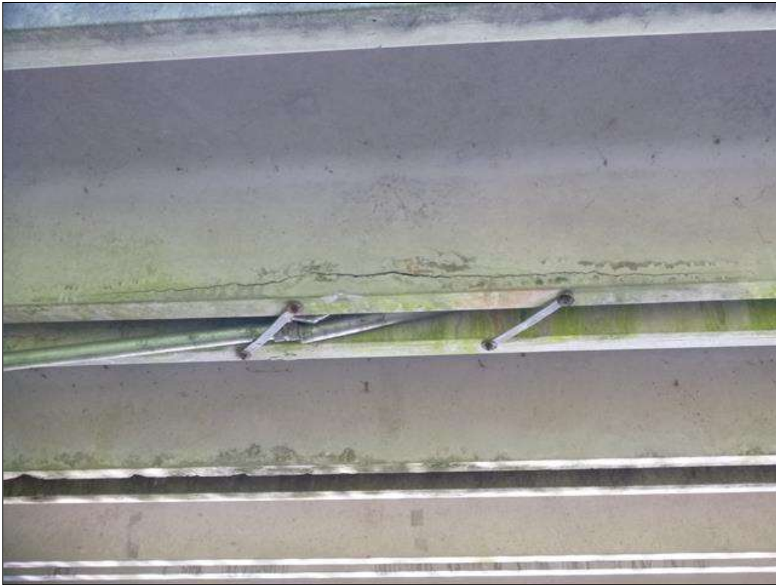
Span 2 Slab 10: left leg at midspan, delamination (4ft x 2in high) with longitudinal crack crack (up to 1/8in)
