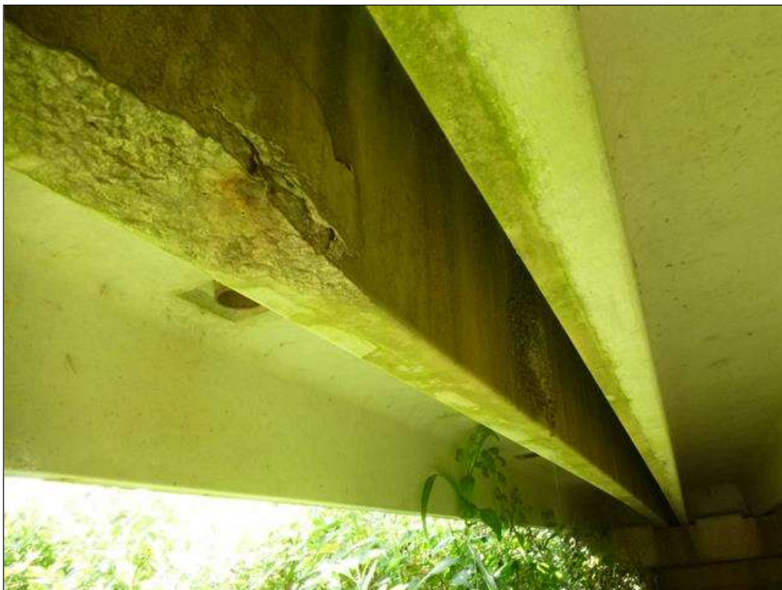
Span 4 Slab 1: right leg near midspan, spall [12in x 8in x 3/4in] with exposed stirrup [no section loss noted]
