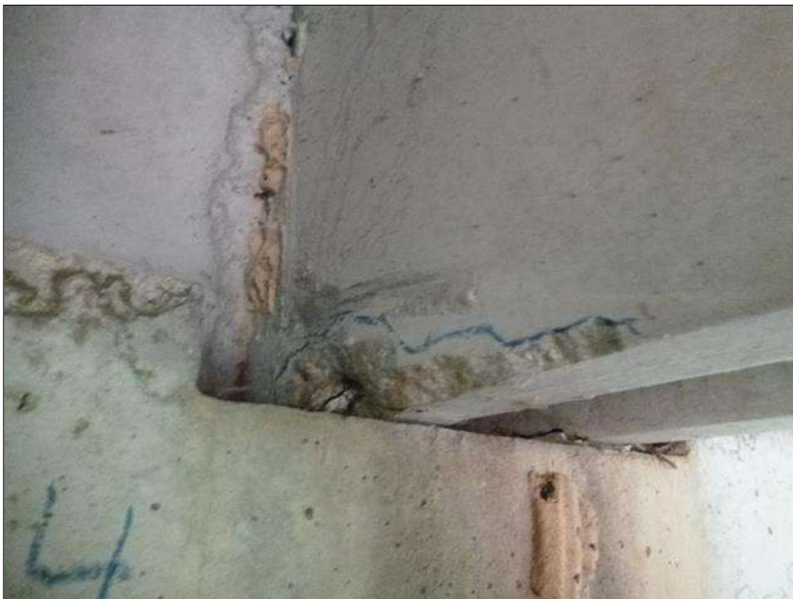
Span 4 Slab 4: (PAR) at far end of both legs, three [3] spalls/delaminations [6in x 6in x 1-1/2in deep] with one exposed strand [section loss up to 10%]
