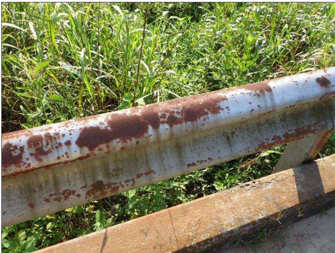
Span 1 Left Bridge Rail: along length of rail, active corrosion with no section loss noted
