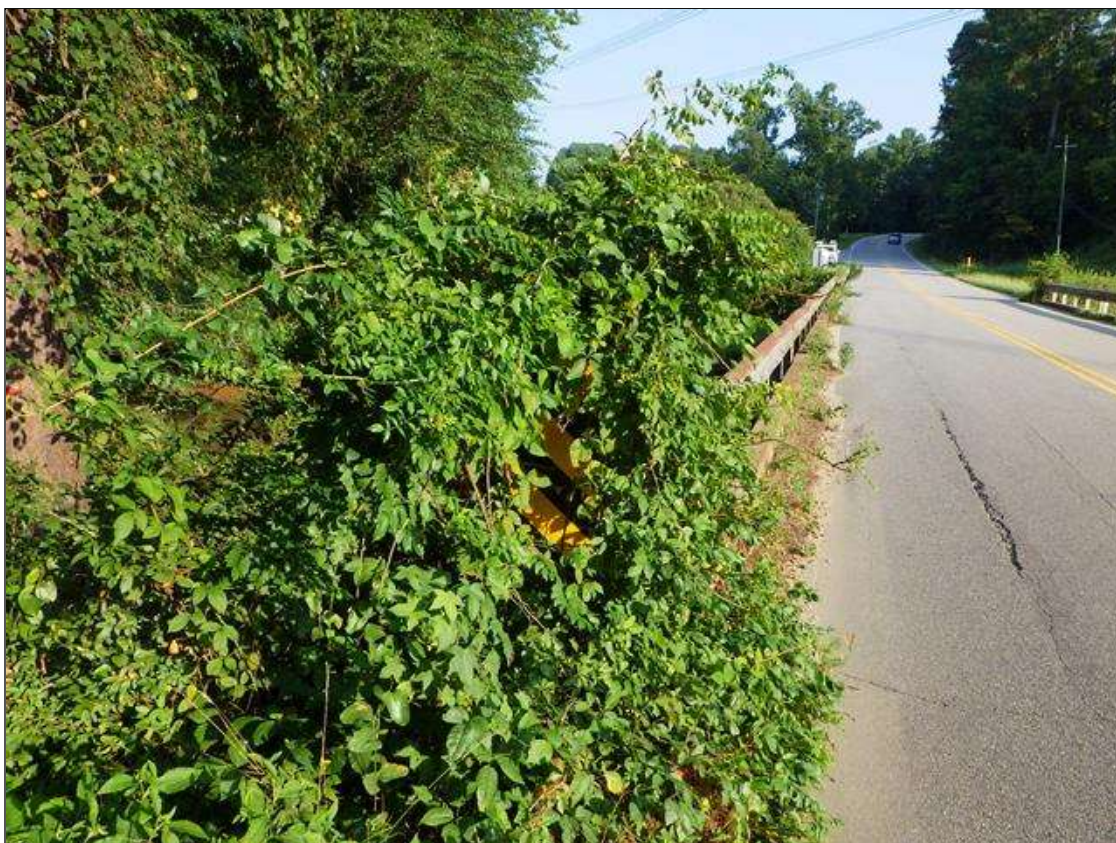
General Comments and Misc. Items: (PAR) northeast delineator covered by vegetation
