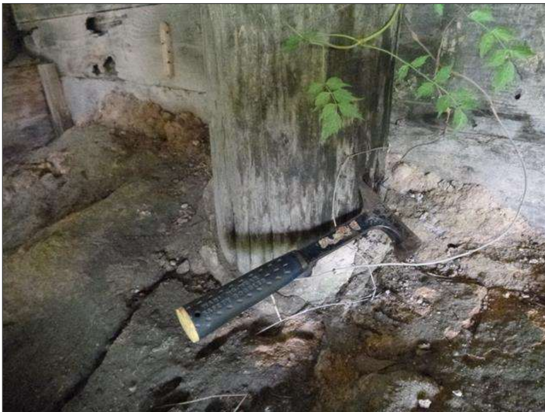
End Bent 1 Pile 3: (PAR) at base of pile, multiple checks [full height x up to 1/4in wide x up to 2in deep], decay [14in x 10in x 3in deep]
