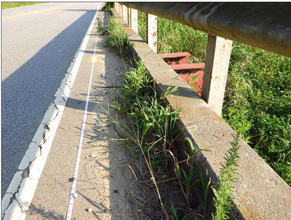
Deck Debris: along both curbs, debris and vegetation (full length x 1ft x up to 3in deep)
