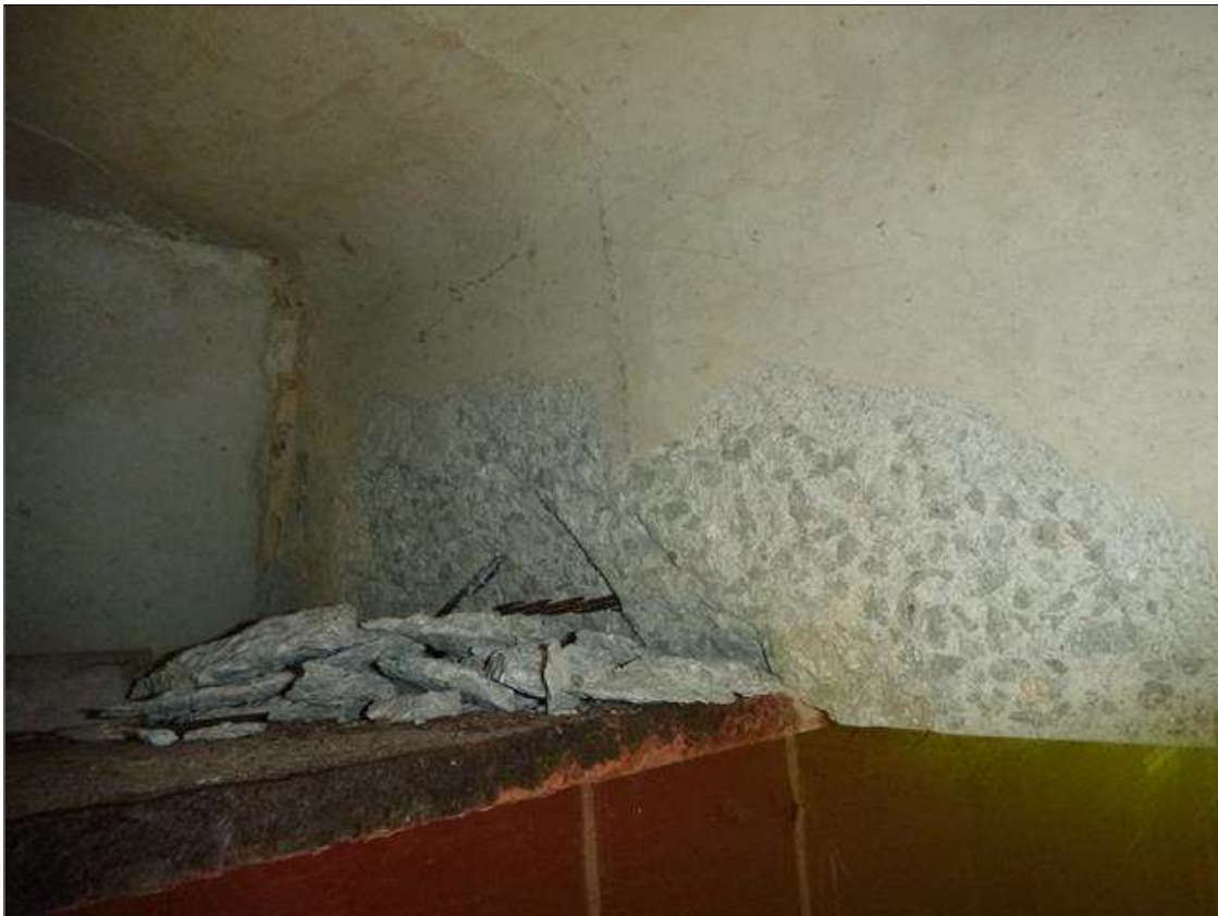
Span 1 Slab 3: (PAR) left and right leg at bent 1, two [2] spalls [up to 12in x 6in x 1in deep] with exposed strand, channel legs crushing and bottom of channel legs sits below top of crutch bent cap
