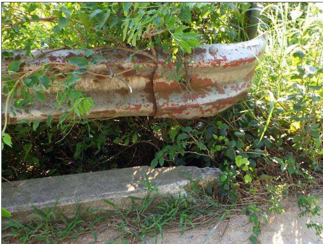
Span 4 Left Bridge Rail: [PAR] rail post 6 is missing
