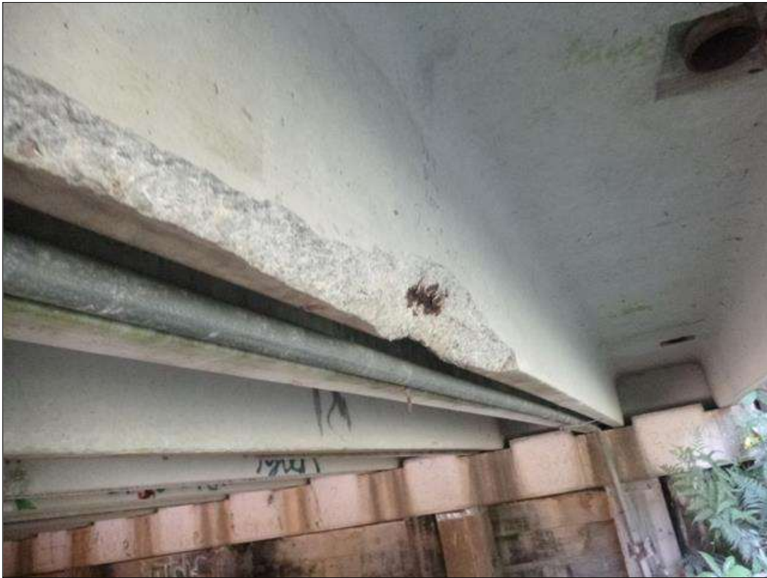
Span 4 Slab 10: [PAR] 5 TOTAL AREAS OF AREAS IN LEFT LEG OF FULL WIDTH X UP TO 6" HIGH SPALLS WITH EXPOSED STRANDS FOR 20' TOTAL (20% SECTION LOSS) (PHOTO 3 OF 4)
