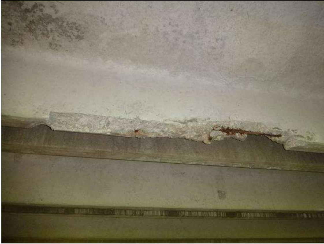
Span 1 Slab 5: (PAR) right leg at midspan, spall (40in x 3in deep) with exposed strand (25% section loss)
