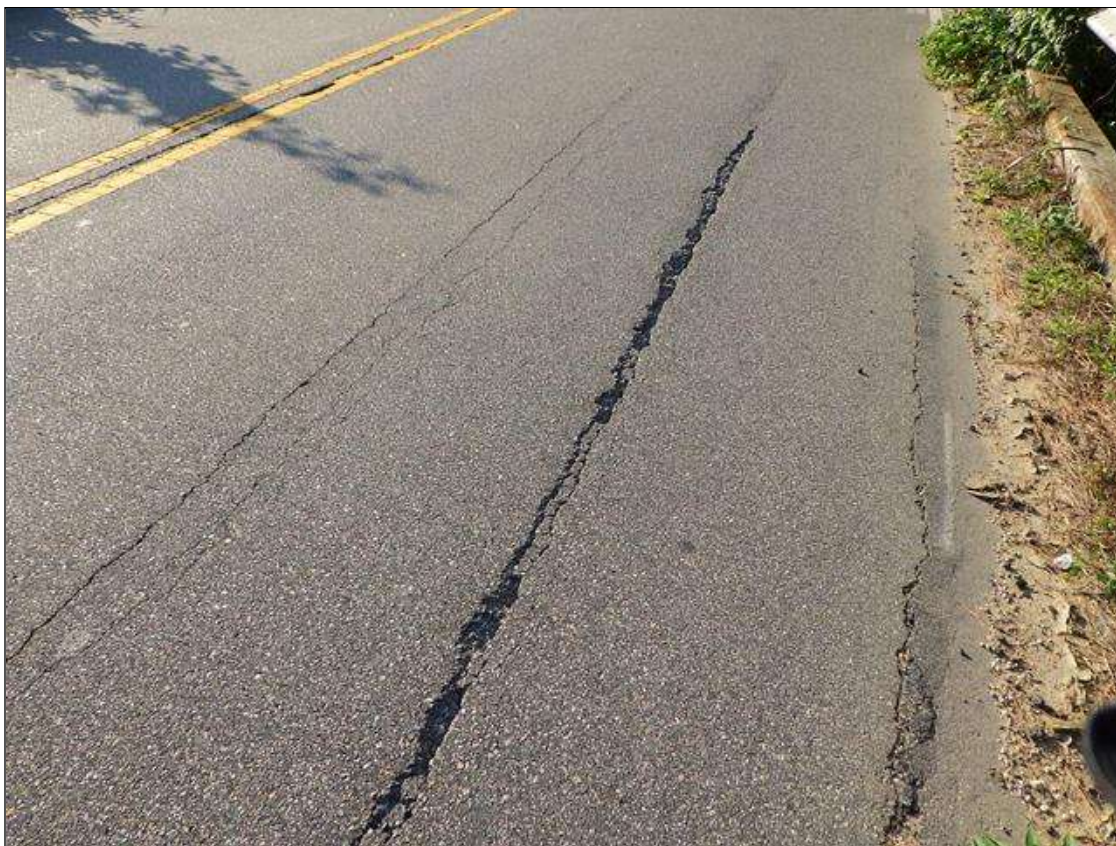
Span 4 Wearing Surface: northbound lane along edge of channels 8 and 9, pothole (20ft x 3in x 1in)
