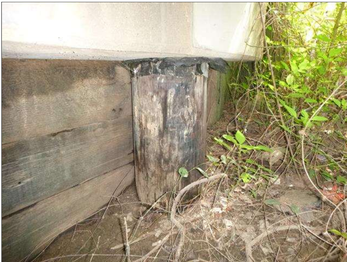
End Bent 1 Pile 1: (PAR) along height of exposed pile, multiple checks [full height x up to 1/8in], pile sounds hollow when hammered
