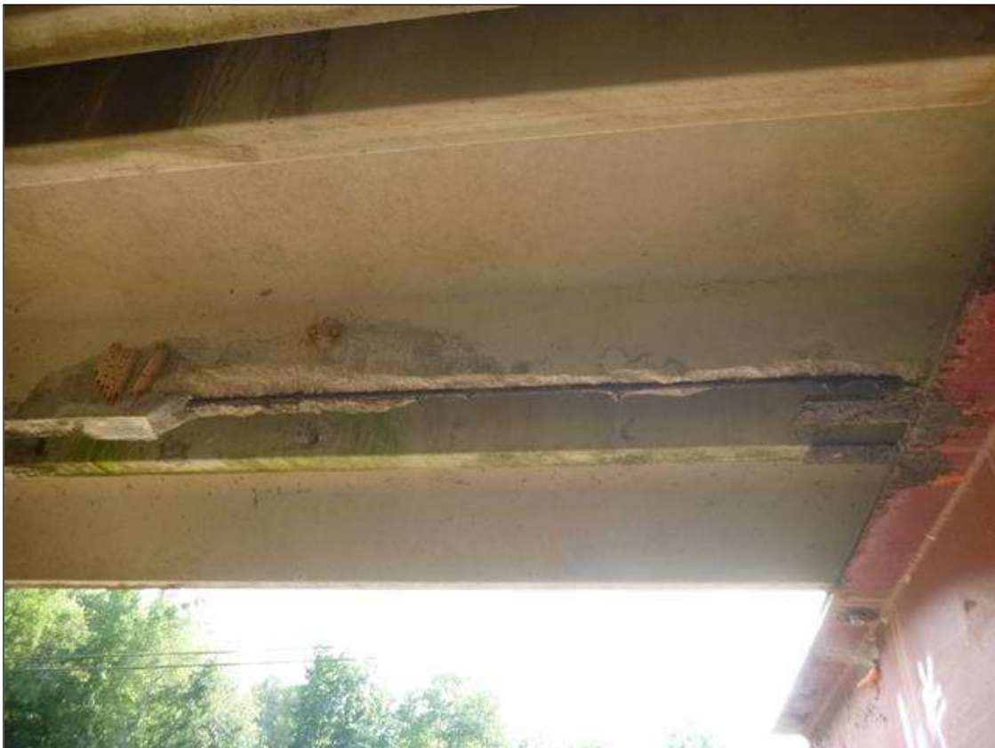
Span 3 Slab 2: [PAR] left leg at bent 3, spall [6ft x full width x 5in], with exposed strand (40% section loss)
