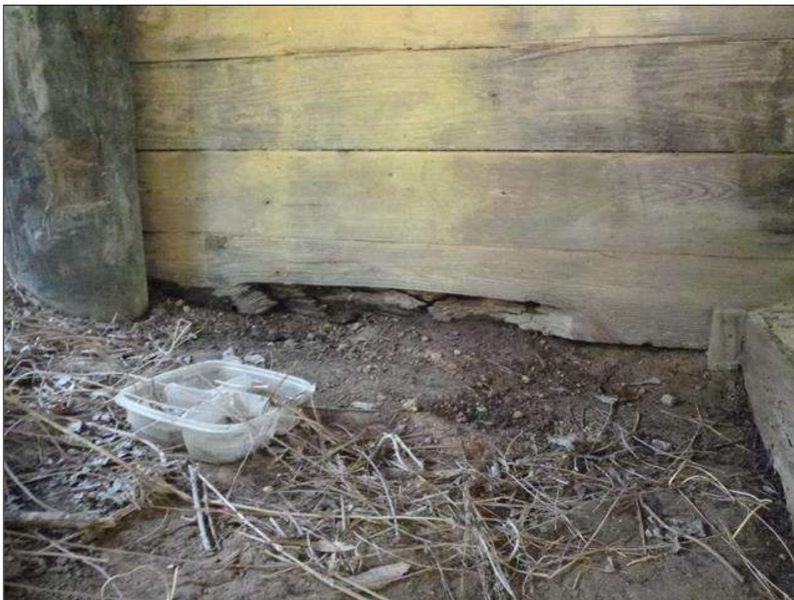
End Bent 2 Abutment: [PAR] between piles 1 and 2, lower board decay [3ft x 4in x full width] with exposed/missing backfill material
