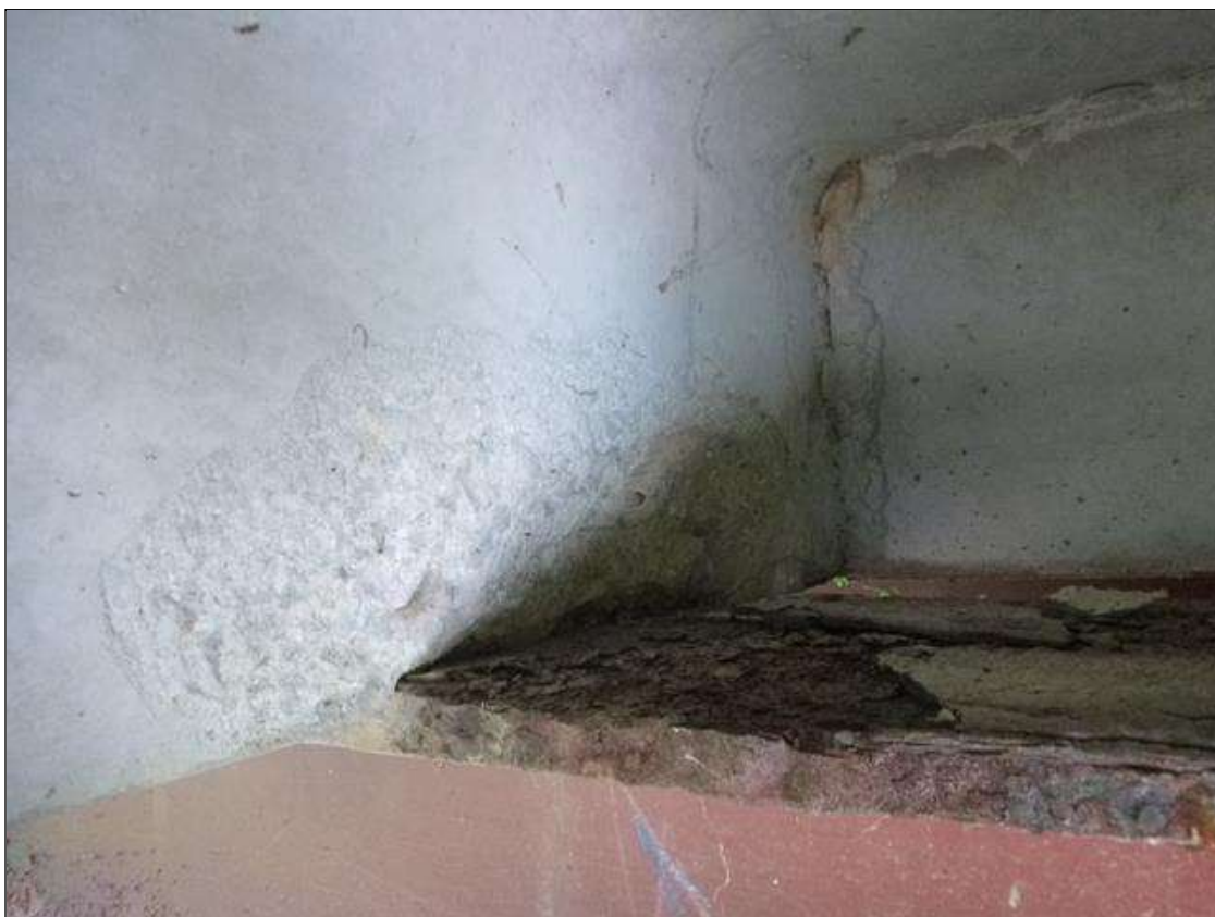
Span 2 Slab 10: left and right leg at bent 1, four [4] spalls [up to 18in x 6in x 1/2in]
