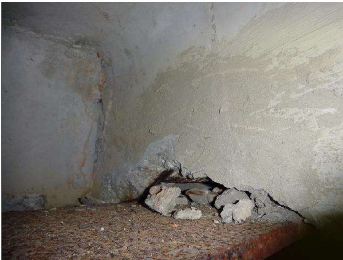
Span 1 Slab 4: (PAR) right leg at bent 1, spalled patched area [12in x full width x 5in high] with exposed strands
