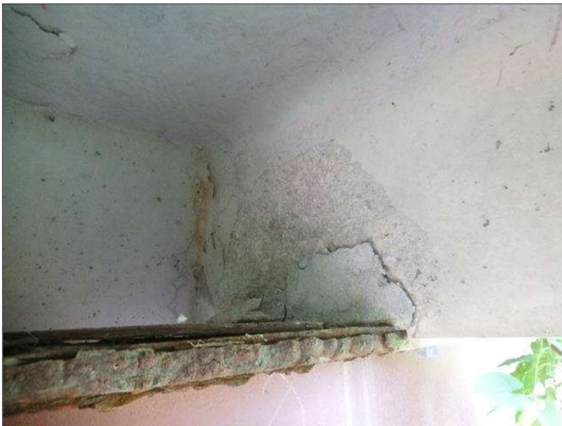
Span 1 Slab 10: right leg at far end over bearing, spall [18in x 9in x 1/2in deep]
