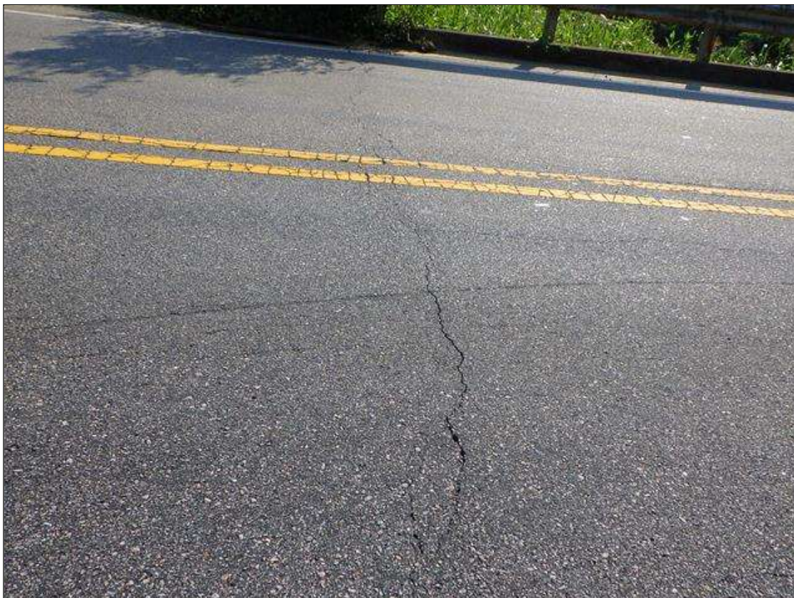
Span 1 Wearing Surface: over end bent 1, transverse crack (full width x up to 1/8in)
