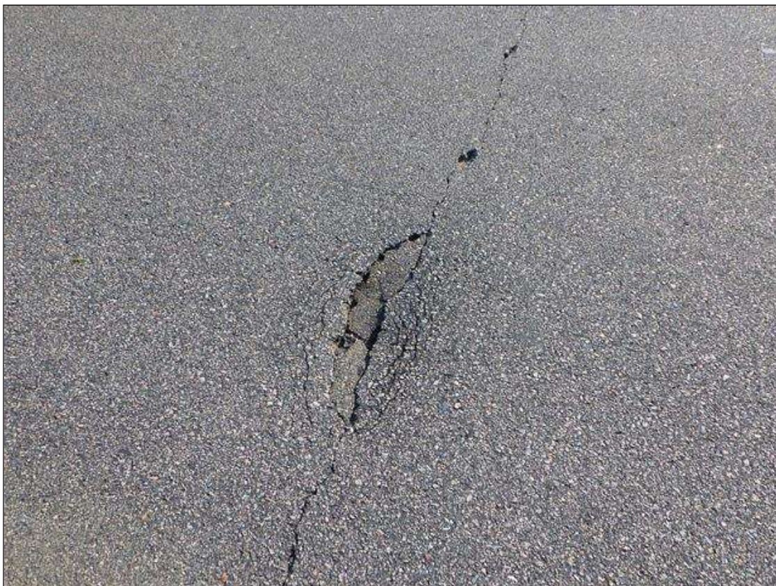
Span 1 Wearing Surface: northbound lane at bent 1, pothole (6in x 20in x up to 1-1/2in deep)
