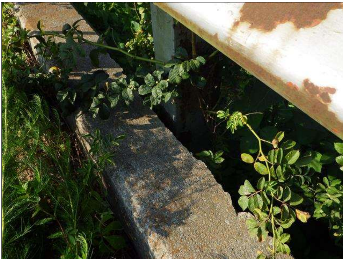
Span 1 Right Bridge Rail: at rail post 2, spall [3ft x 10in x 3in deep]
