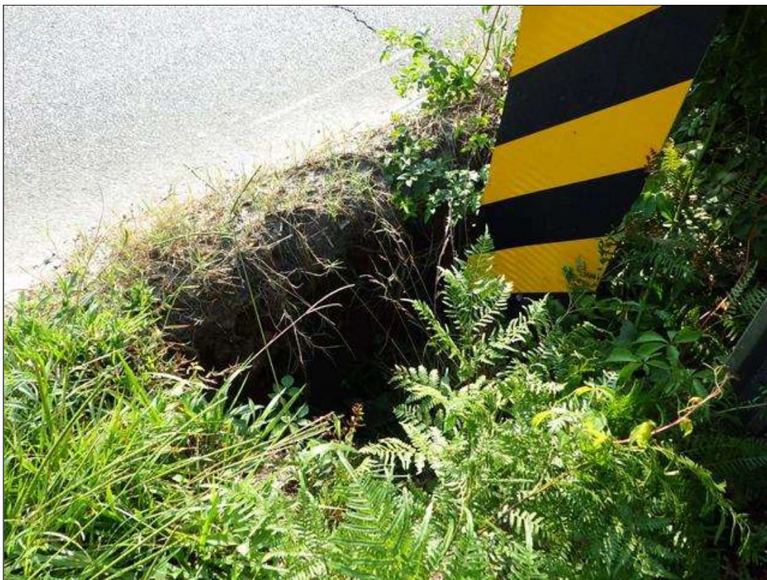
General Comments and Misc. Items: (PAR) southeast corner of bridge adjacent to roadway, erosion hole (3ft long x 2.5ft wide x up to 4ft deep) up to 1ft of undermining of roadway
