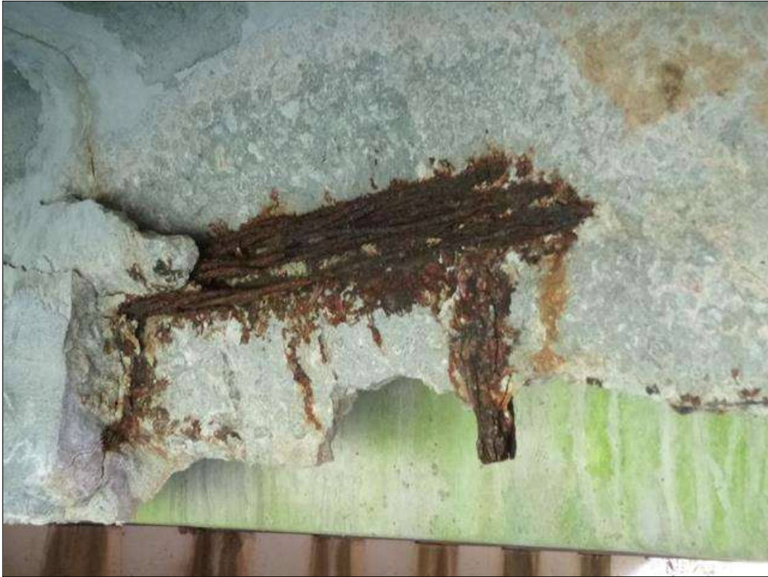
Span 1 Slab 10: [PAR] left leg at midspan, spall/delamination, [11ft x full width of leg x 11in high] with four [4] exposed prestressed strands, three [3] of the exposed strands have failed with remaining one [1] strand exhibiting section loss [up to 40%] (photo 2 of 2)
