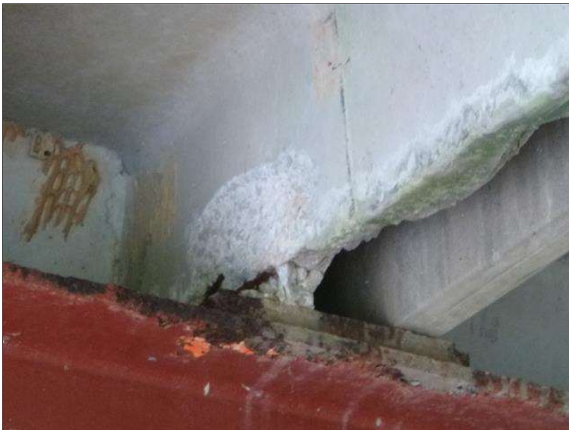
Span 3 Slab 5: (PAR) right leg at bent 3, spall [6in x 4in x full width], with exposed strand
