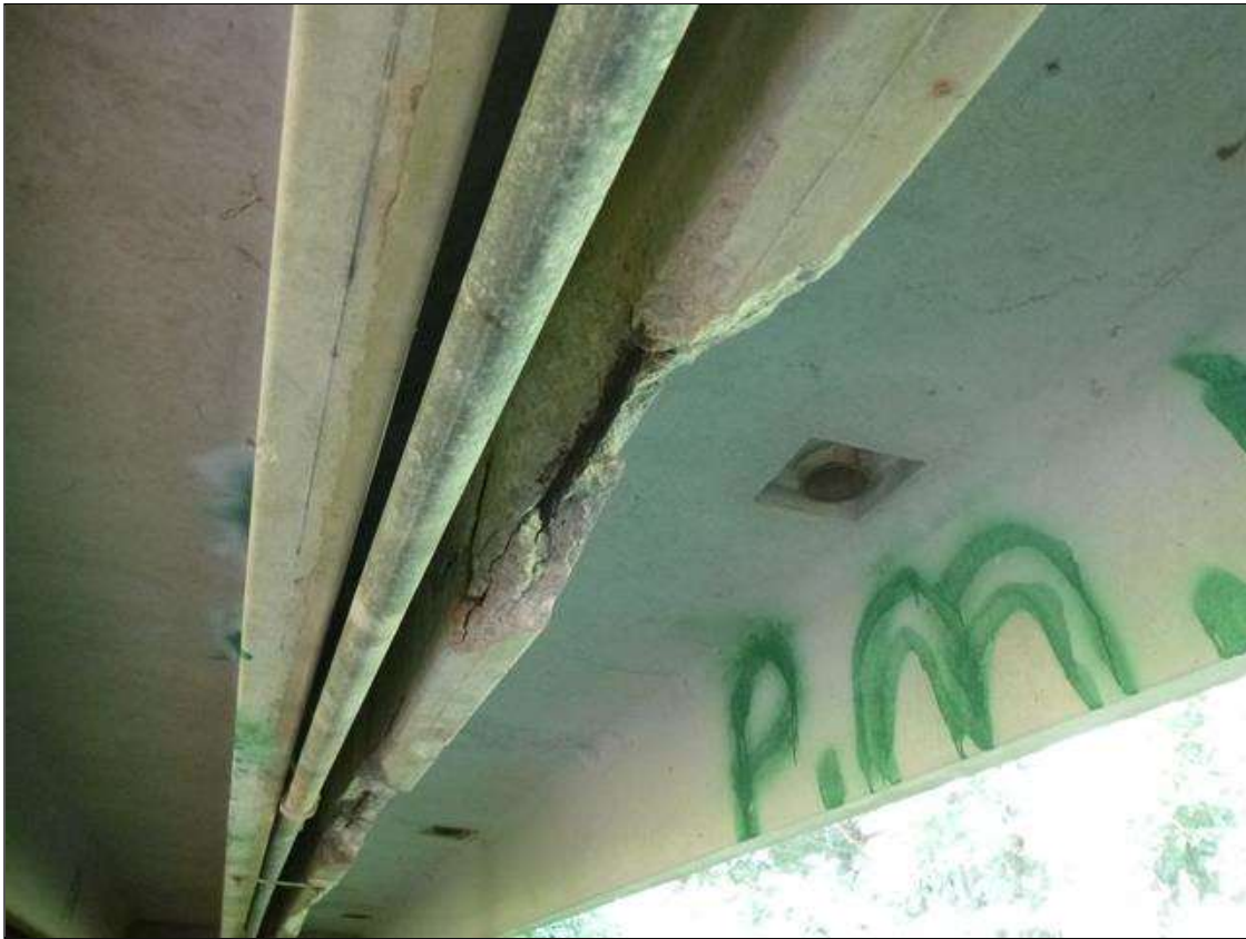
Span 4 Slab 10: [PAR] 5 TOTAL AREAS OF AREAS IN LEFT LEG OF FULL WIDTH X UP TO 6" HIGH SPALLS WITH EXPOSED STRANDS FOR 20' TOTAL (20% SECTION LOSS) (PHOTO 1 OF 4)
