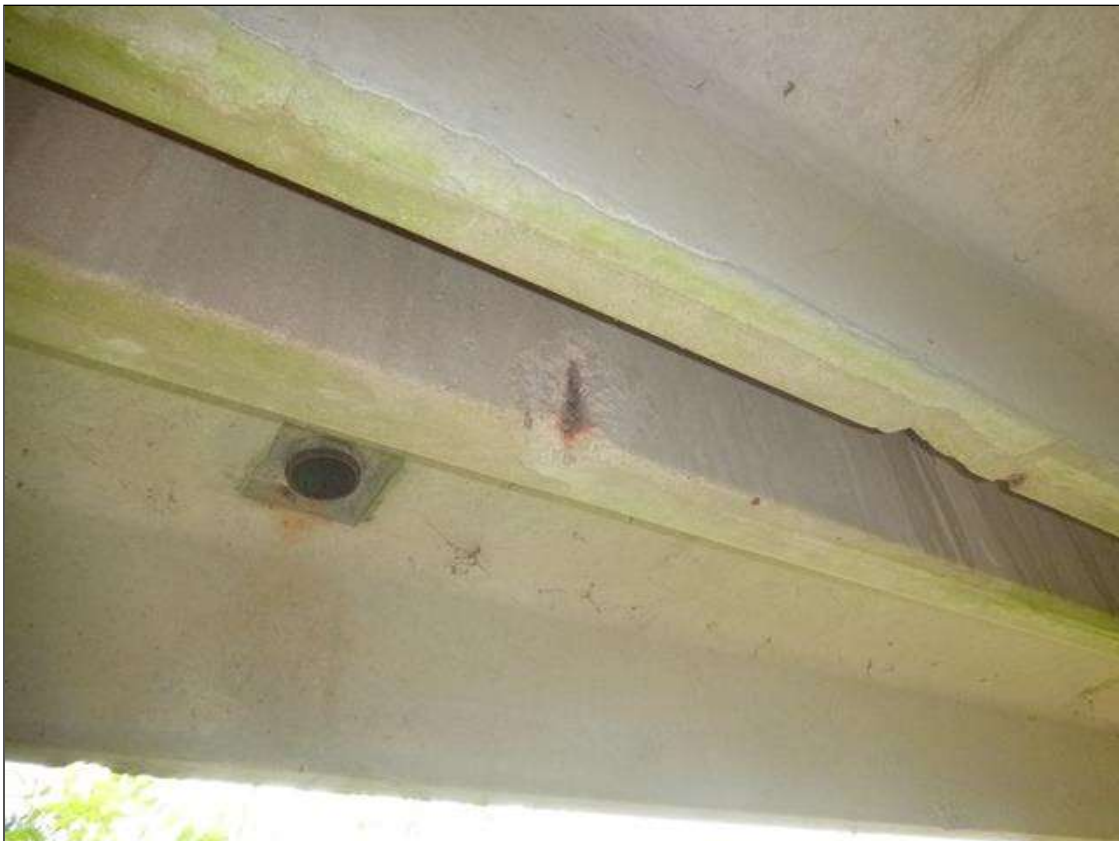
Span 1 Slab 1: left and right leg near midspan, multiple spalls/delaminations [up to 5in x 4in x 3/4in deep] with two exposed stirrups [no section loss noted]
