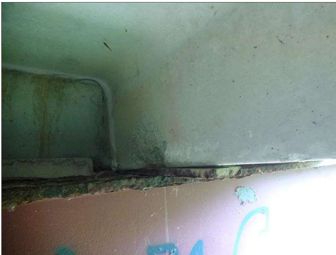
Span 4 Slab 2: left leg at bent 3, spall [6in x 6in x 1/2in deep]
