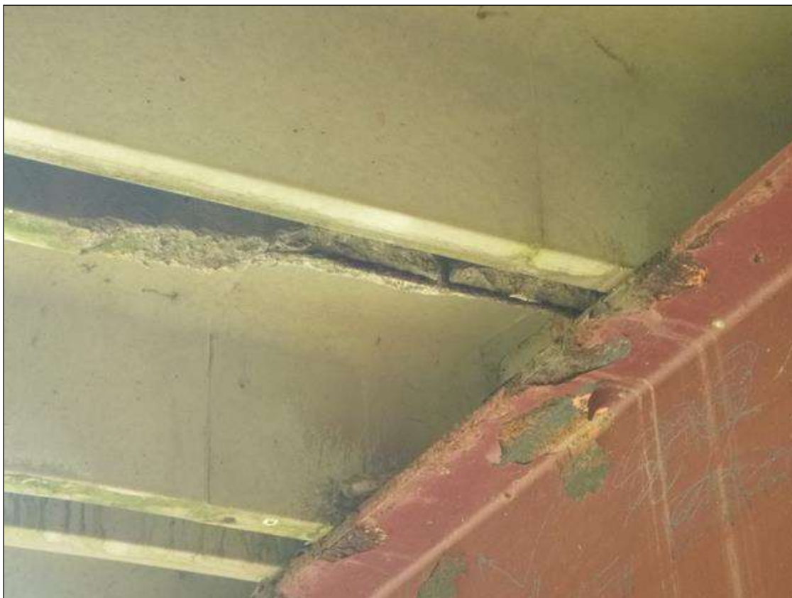
Span 2 Slab 2: [PAR] left and right leg at bent 2, two [2] spalls/delaminations [up to 36in x 6in x full width], with two [2] exposed stirrups [no section loss noted] and exposed strand [section loss up to 20%]
