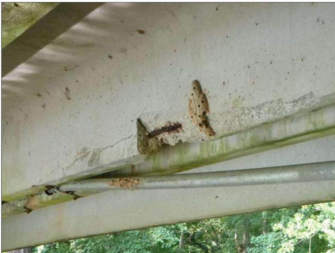
Span 2 Slab 9: [PAR] right leg 12ft from bent 1, spall/delamination [6ft x 3in x full width] with exposed strand (25% section loss)
