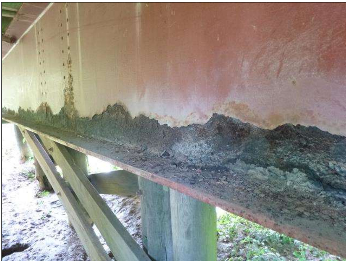
Span 1 Crutch Bent 1 Cap 1: along length of cap at lower web and top flange, corrosion with section loss [ <1/16 in] with adjacent spot rust
