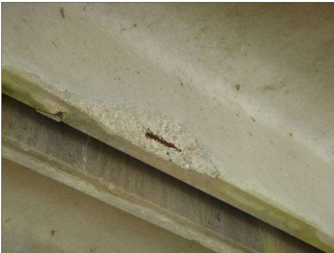
Span 3 Slab 2: (PAR) right leg at midspan, spall (20in x 5in x 3/4in) with exposed rusted strand
