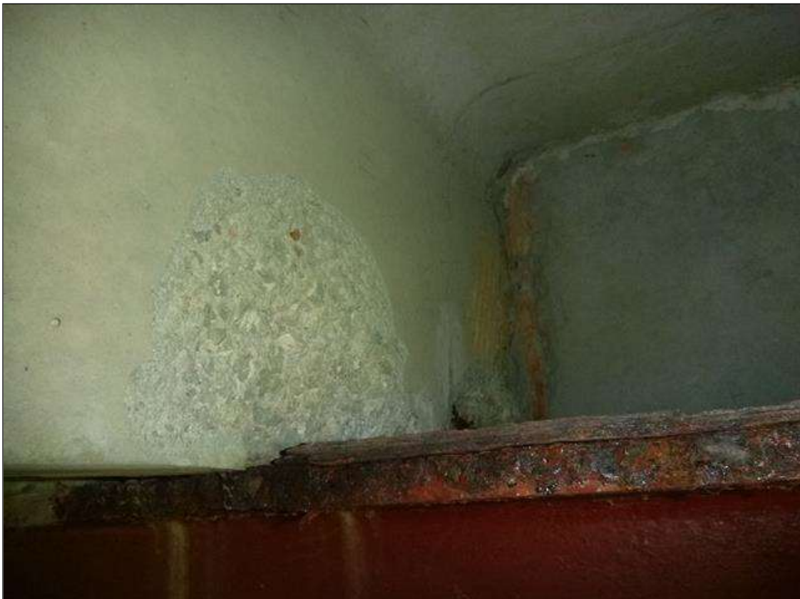
Span 1 Slab 9: left leg at far end, two [2] spalls [up to 4in diameter x 1in deep] with one [1] exposed stirrup [loss < 1/16in]
