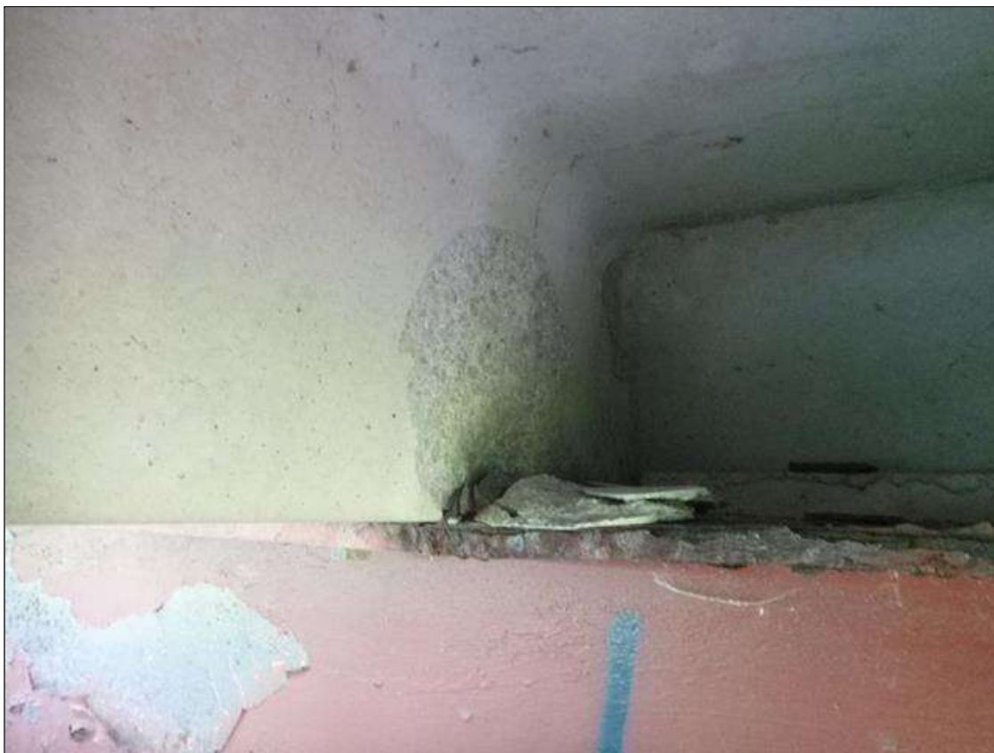
Span 4 Slab 10: right leg at bent 3, spall [10in x 4in x 3/4in deep]
