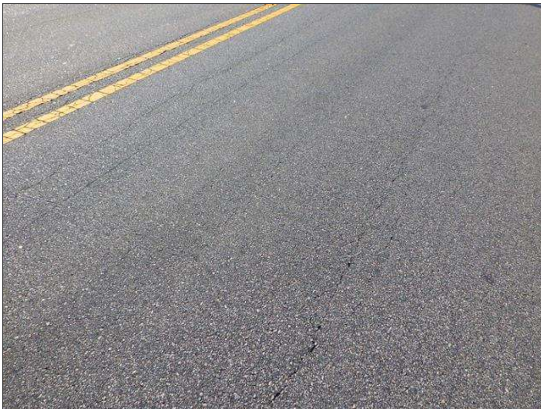
Span 1 Wearing Surface: along edges of channels, (5) longitudinal cracks (full length x 1/16in)
