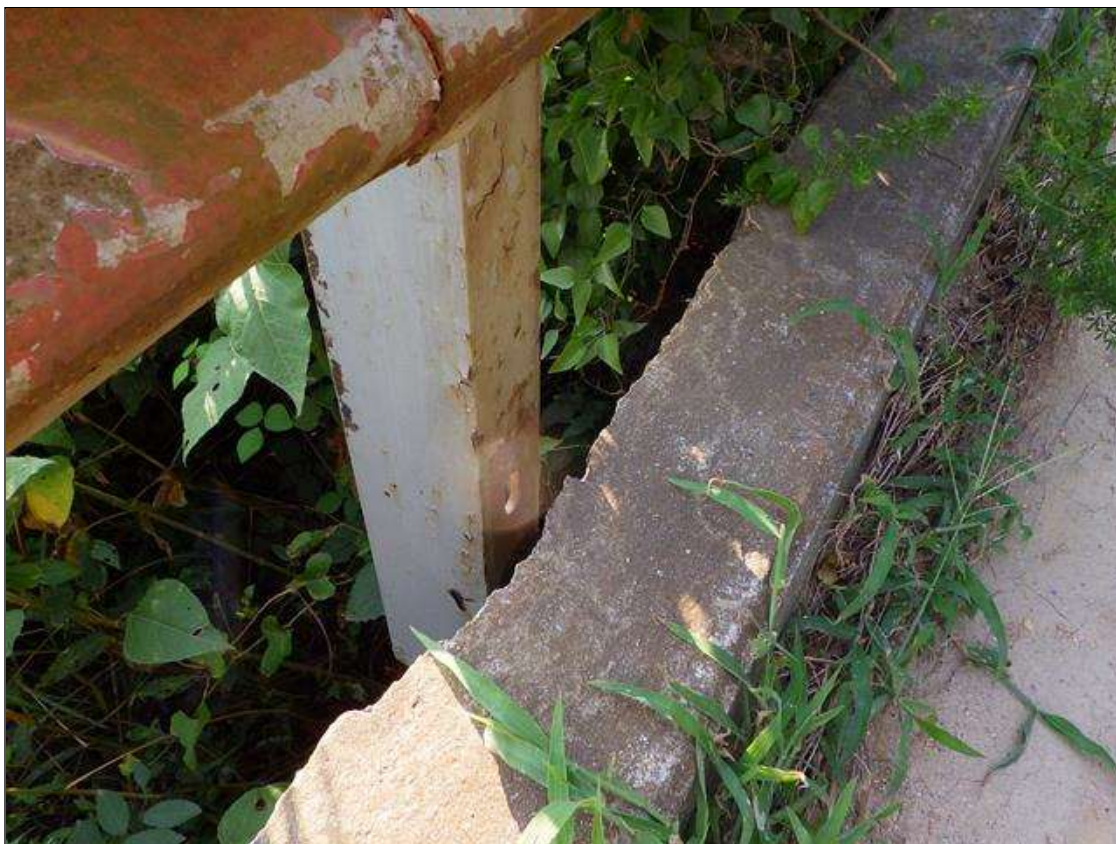
Span 4 Left Bridge Rail: (PAR) at rail posts 3,4 & 5, delamination/spall [up to 3ft x 11in x 3in deep] allowing excessive deflection of rail
