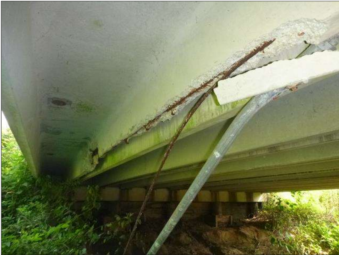
Span 1 Slab 10: [PAR] left leg at midspan, spall/delamination, [11ft x full width of leg x 11in high] with four [4] exposed prestressed strands, three [3] of the exposed strands have failed with remaining one [1] strand exhibiting section loss [up to 40%] (photo 1 of 2)
