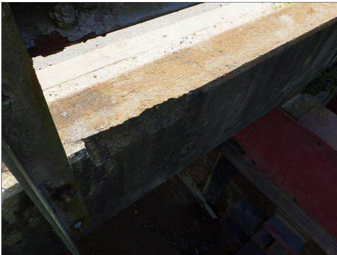
Span 2 Right Bridge Rail: at rail post 5, delamination/spall [2ft x 8in x 3in deep]
