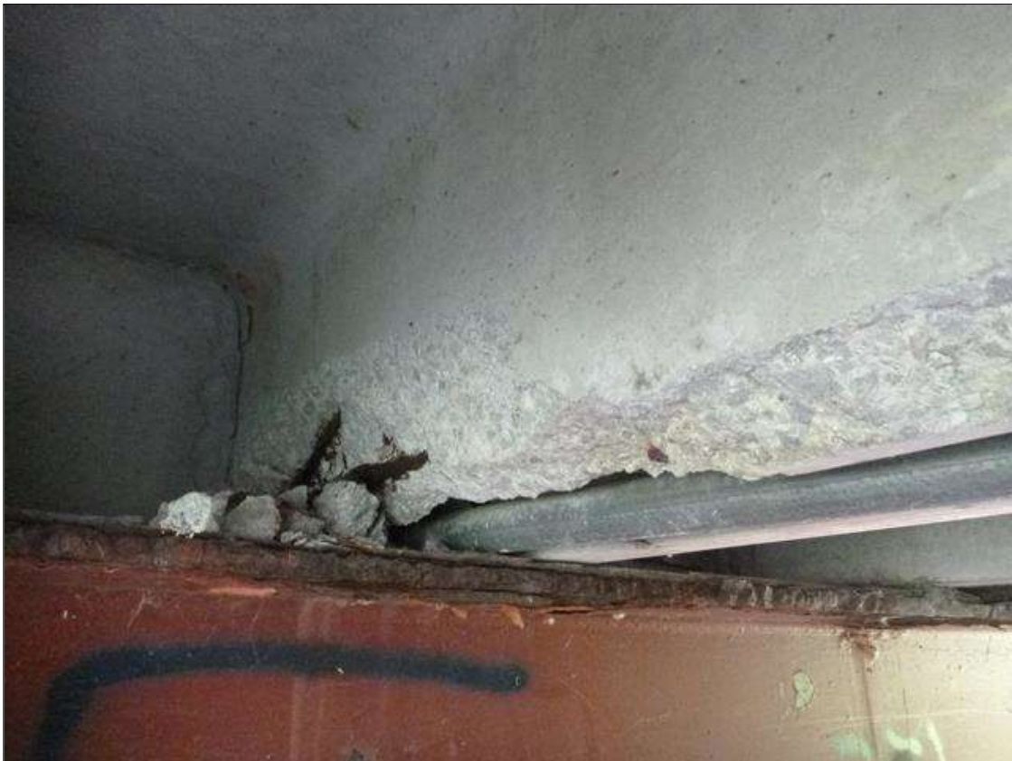
Span 4 Slab 10: [PAR] 5 TOTAL AREAS OF AREAS IN LEFT LEG OF FULL WIDTH X UP TO 6" HIGH SPALLS WITH EXPOSED STRANDS FOR 20' TOTAL (20% SECTION LOSS) (PHOTO 4 OF 4)
