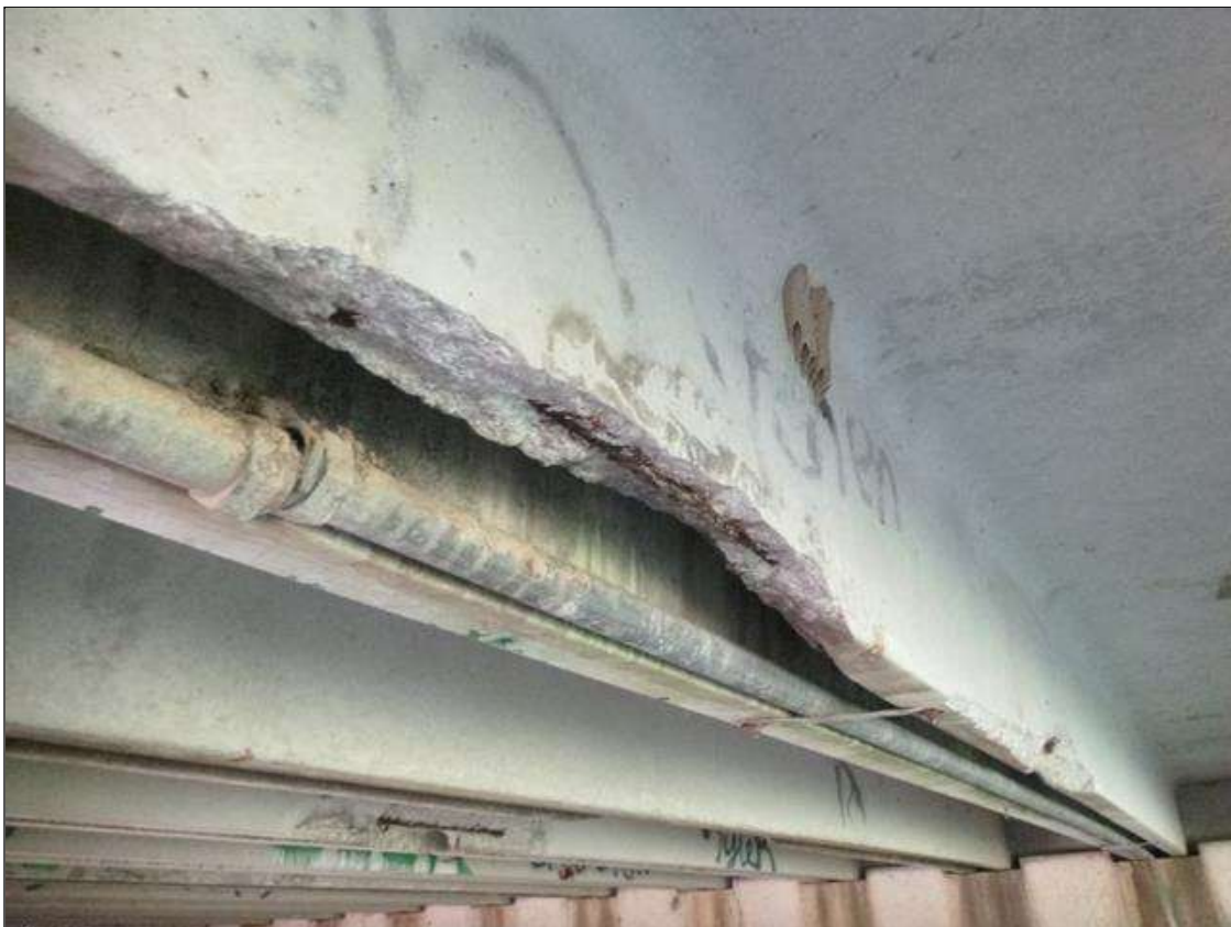
Span 4 Slab 10: [PAR] 5 TOTAL AREAS OF AREAS IN LEFT LEG OF FULL WIDTH X UP TO 6" HIGH SPALLS WITH EXPOSED STRANDS FOR 20' TOTAL (20% SECTION LOSS) (PHOTO 2 OF 4)
