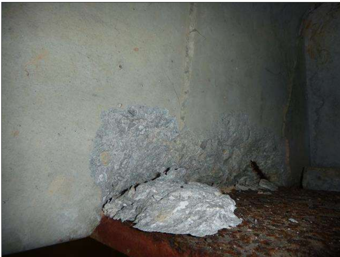
Span 1 Slab 4: left leg at bent 1, two [2] spalls [up to 12in x 4in x 1in deep]
