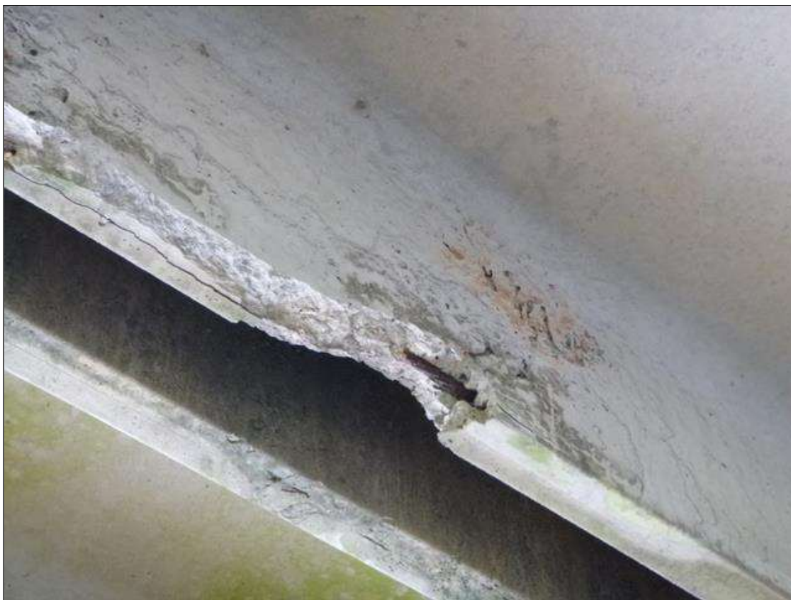
Span 3 Slab 6: [PAR] left leg at far third, spall [2ft x 5in] with exposed strand
