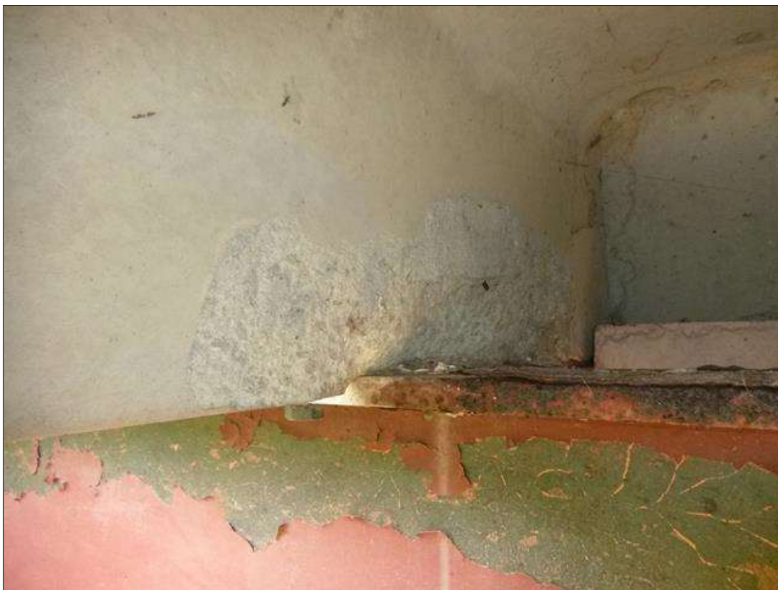
Span 1 Slab 1: (PAR) left and right leg at bent 1, four [4] spalls/delaminations [up to 12in x 5in x 1in deep] with loss of bearing area
