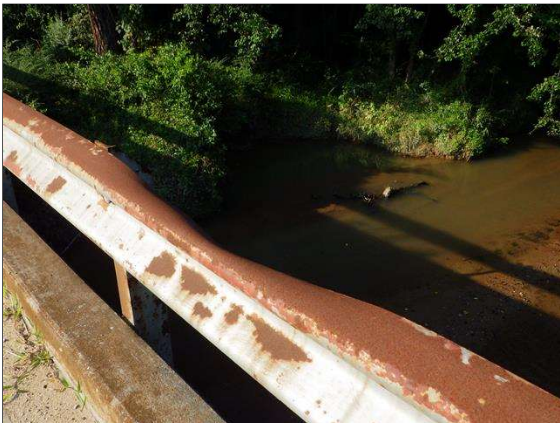
Span 3 Right Bridge Rail: along length of rail at top, three [3] areas of impact damage [up to 3ft x 3in]
