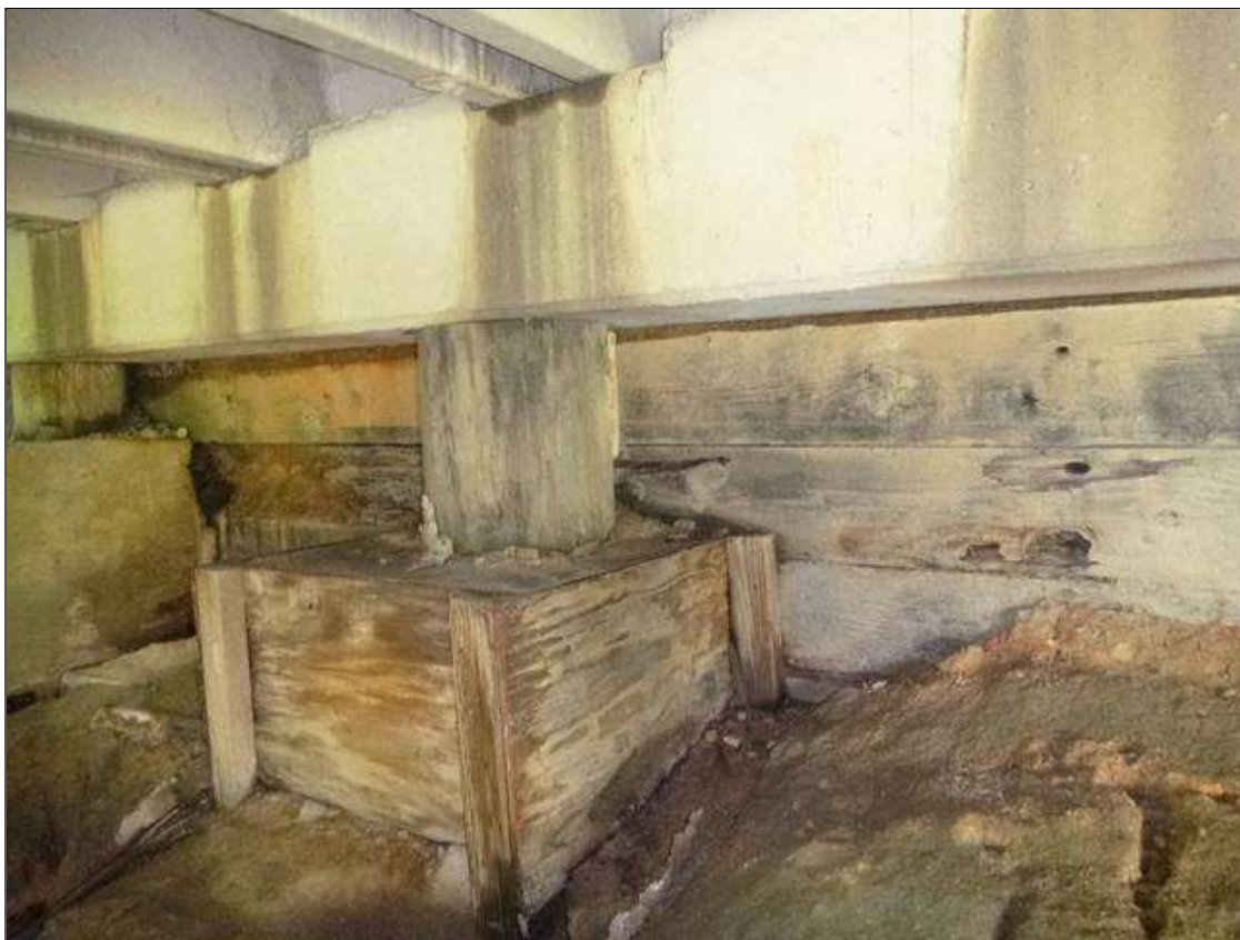
End Bent 1 Abutment: [PAR] between piles 3 and 5 second bulkhead board below cap, decay [10ft x up to full height x full width] with fill exposed
