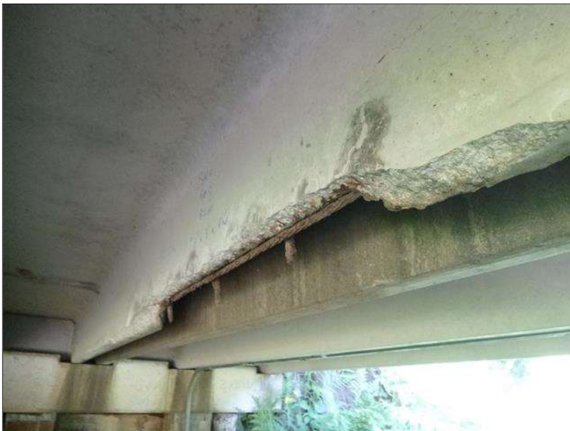
Span 4 Slab 8: [PAR] right leg at far third, spall [4ft x 3in x full width] with exposed strand
