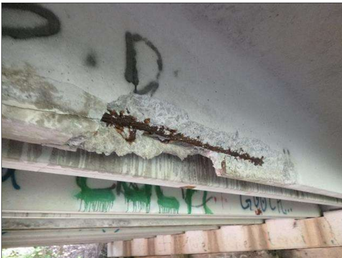
Span 4 Slab 8: (PAR) left leg at far third, spall/delamination [36in x 3in x 2in deep] with exposed rusted strand
