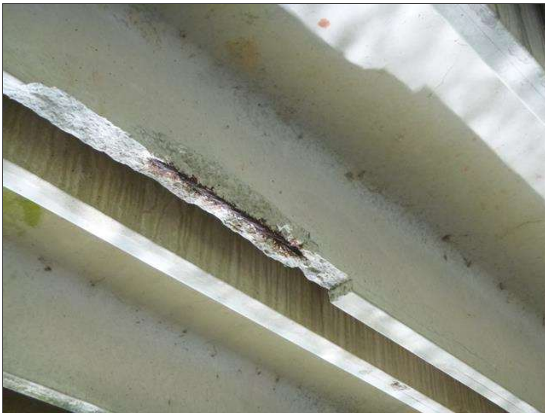
Span 2 Slab 7: [PAR] left leg near midspan, spall/delamination [30in x 4in x full width], with exposed strand [section loss up to 30%]
