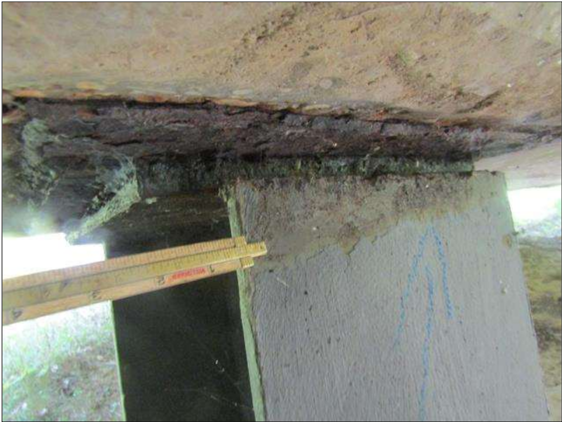
PILES NOT CENTERED ON PLATES ARE MISALIGNED
