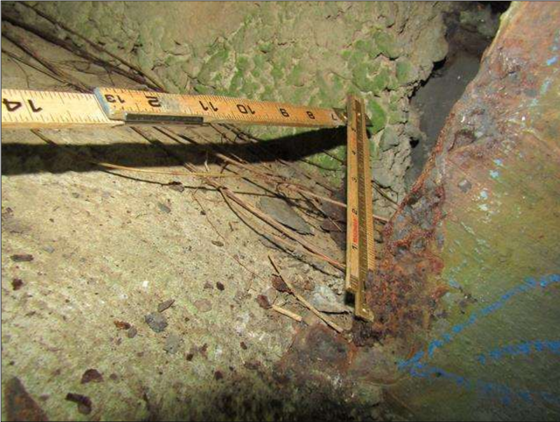
End Bent 1 Pile 6: RUST SCALE WITH REMAINING STEEL DOWN TO KNIFE EDGE ON EAST SIDE FRONT FLANGE UP 5" HIGH ABOVE FOOTING X 2" WIDE WITH EDGE BREAKING OFF/ PAR
