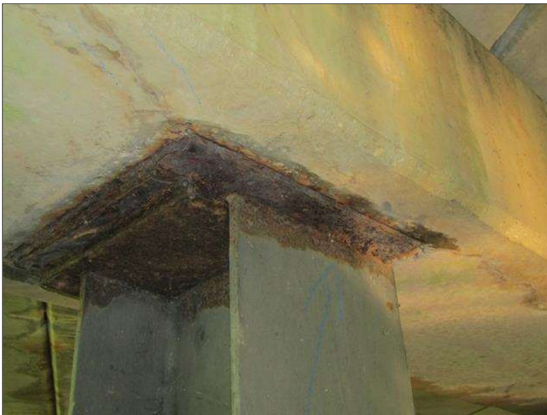
Bent 2 Pile 2: SURFACE AND RUST SCALE ON TOP OF PILE AND PLATE
