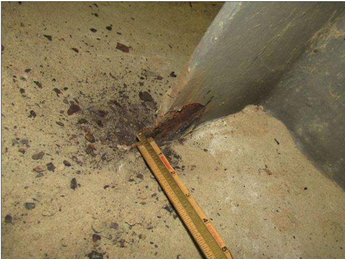
Bent 1 Pile 4: RUST SCALE ON PILE PLATE WITH SURFACE RUST ON TOP AND RUST SCALE ON BOTTOM OF FLANGE ON EAST SIDE ON SOUTH FACE UP 3" X 2" WIDE WITH 1/4" STEEL REMAINING ON 1/2" FLANGE/PAR
