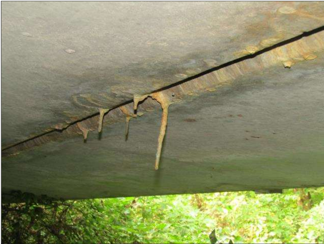
Span 1 Slab 1: EFFLO BUILT UP ON BOTTOM FROM BETWEEN SLABS
