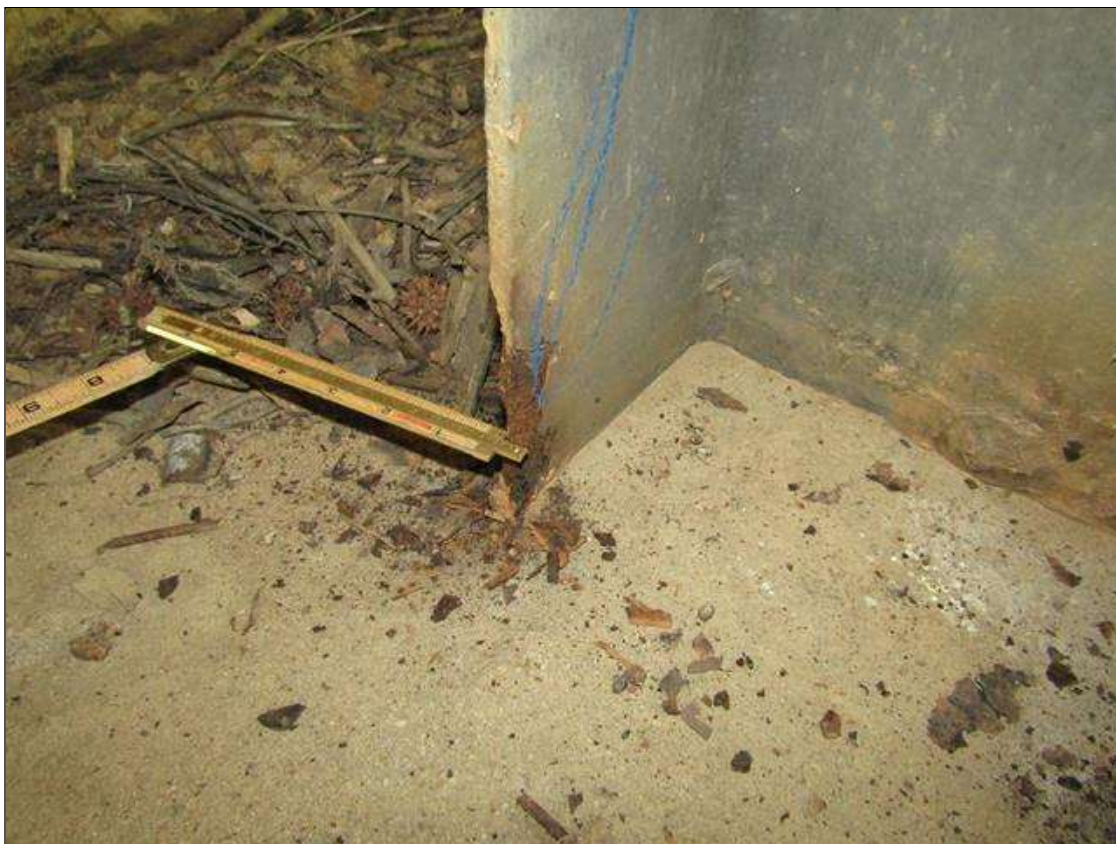
Bent 2 Pile 5: RUST SCALE ON BOTTOM OF NORTH FLANGE ON WEST SIDE UP 2" X 1" WIDE WITH 1/4" STEEL REMAINING ON 1/2" FLANGE/PAR
