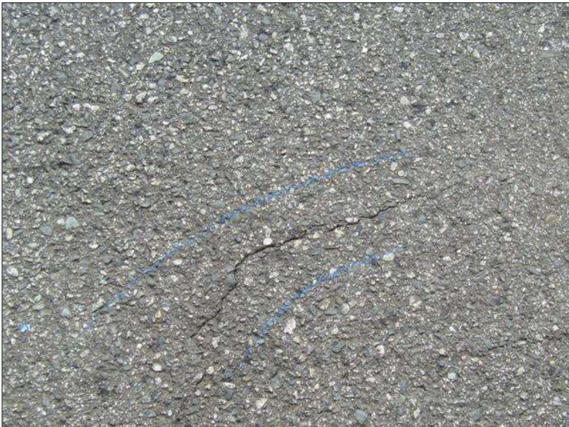
Span 3 Wearing Surface: LONGITUDINAL CRACKS 1/16" WIDE NEAR END BENT 2
