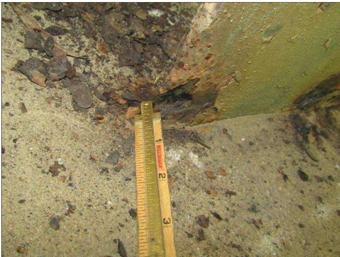
Bent 2 Pile 4: RUST SCALE ON BOTTOM OF SOUTH FLANGE ON WEST SIDE UP 4" X 2" WIDE WITH 1/8" STEEL REMAINING ON 1/2" FLANGE/PAR
