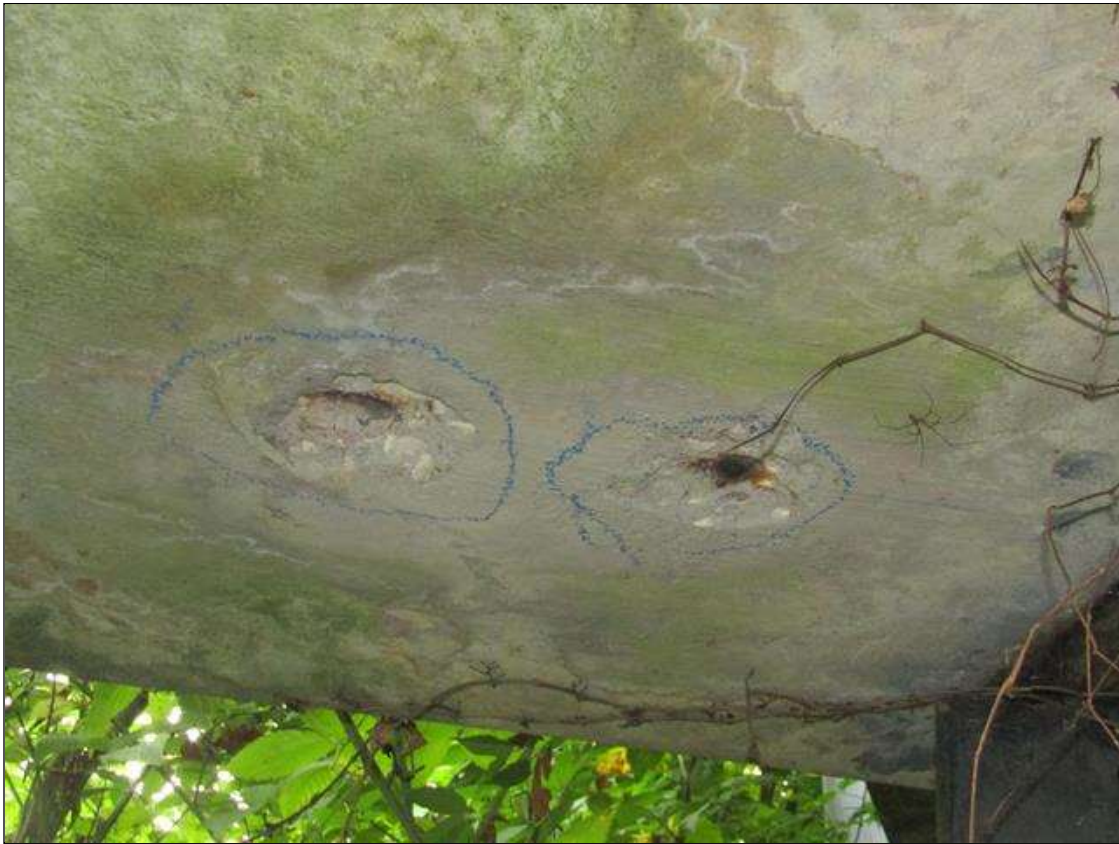
Bent 1 Cap 1: SPALLS ON BOTTOM AT EAST END AND ON BOTTOM BETWEEN PILES 6 -7 UP TO 4" DIAMETER X 1/2" DEEP WITH STEEL EXPOSED
