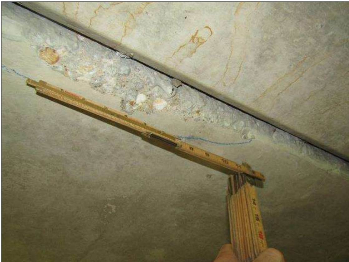
Span 3 Slab 5: SPALL ON RIGHT BOTTOM EDGE 10" LONG X 2" WIDE X 1/2" DEEP NEAR MID SPAN
