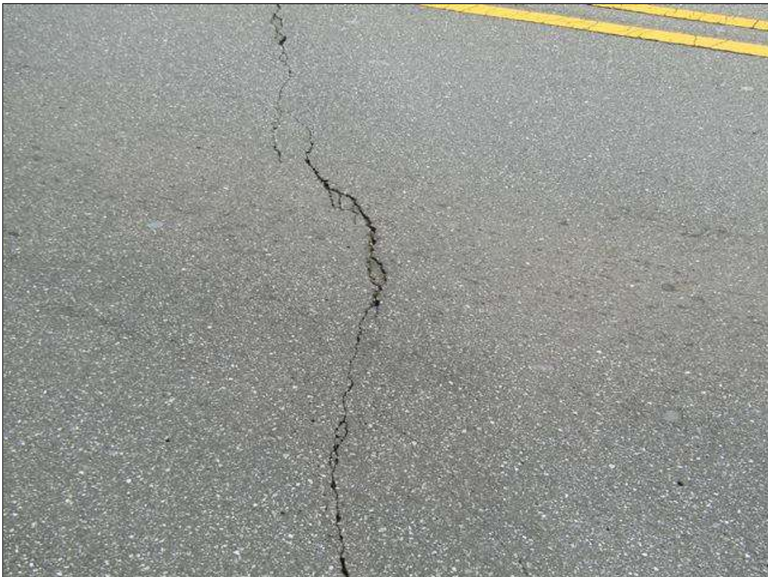
Span 1 Wearing Surface: TRANSVERSE CRACKING OVER END BENT 1 UP TO 1" WIDE
