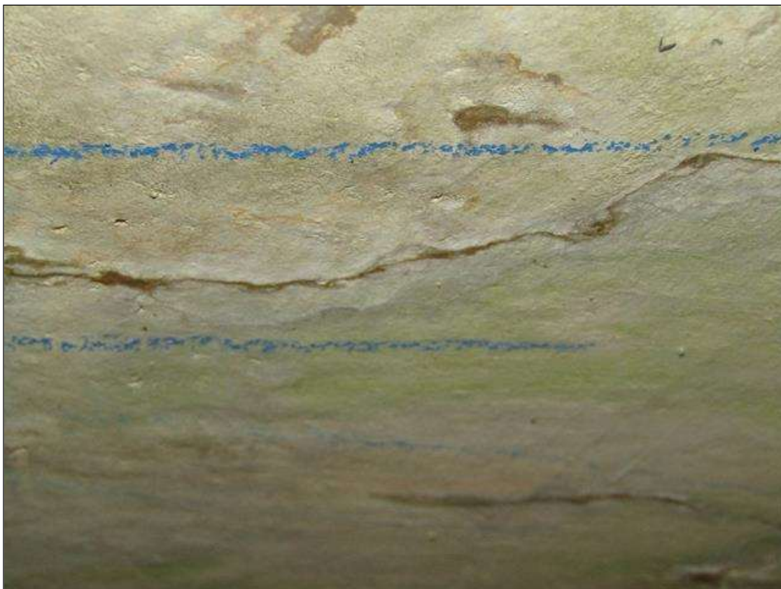
Bent 1 Cap 1: LONGITUDINAL CRACK ON BOTTOM 1/64" WIDE BETWEEN PILES 1-3
