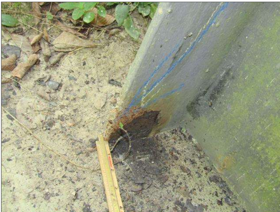
Bent 2 Pile 1: RUST SCALE ON TOP OF PLATE WITH SURFACE RUST ON TOP OF PILE, RUST SCALE ON BOTTOM WEST NORTH FLANGE WITH 1/4" STEEL REMAINING ON 1/2" FLANGE AREA STARTING AT BOTTOM 4" HIGH X 3" WIDE/PM
