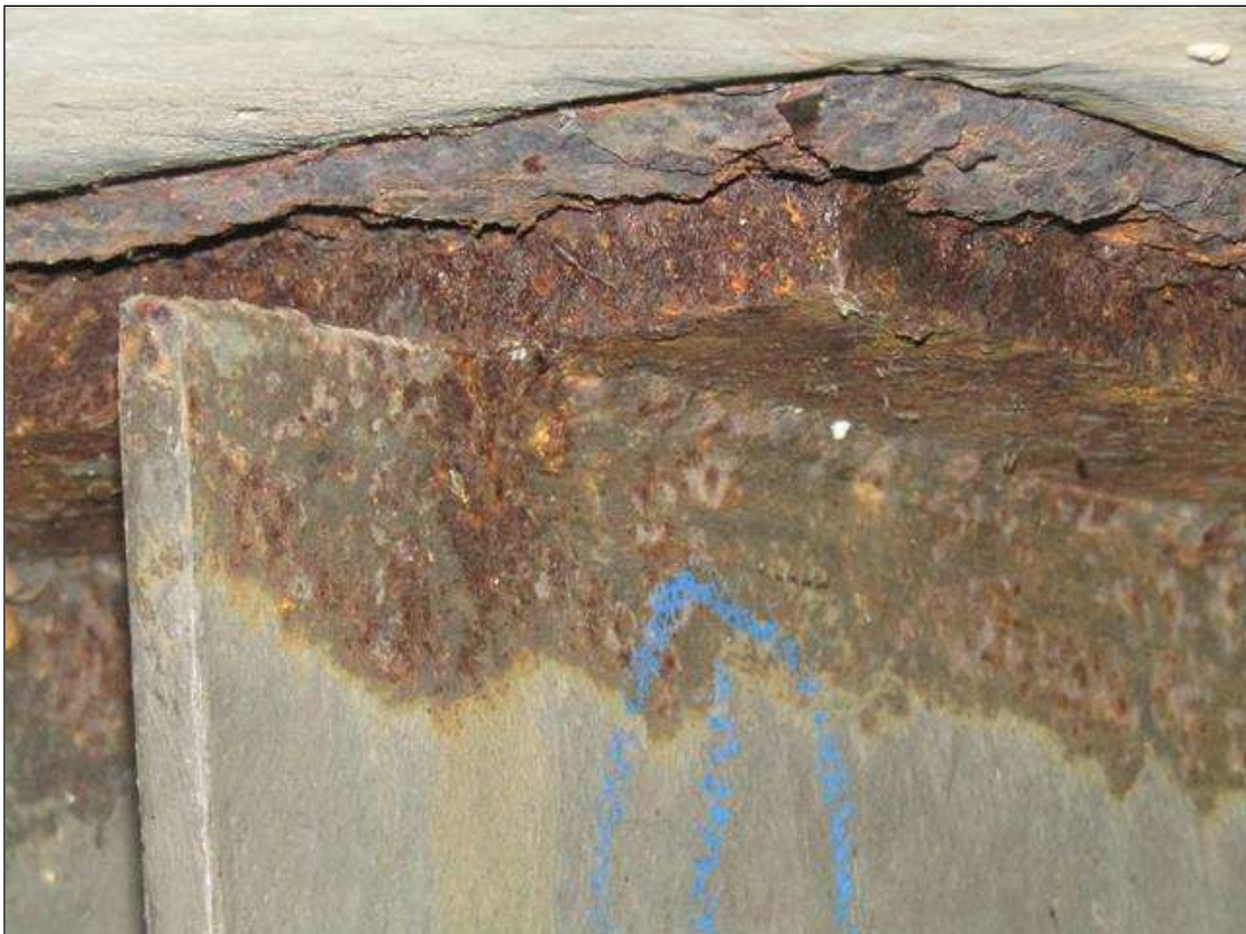
Bent 1 Pile 1: RUST SCALE ON PILE PLATE WITH SURFACE RUST ON TOP
