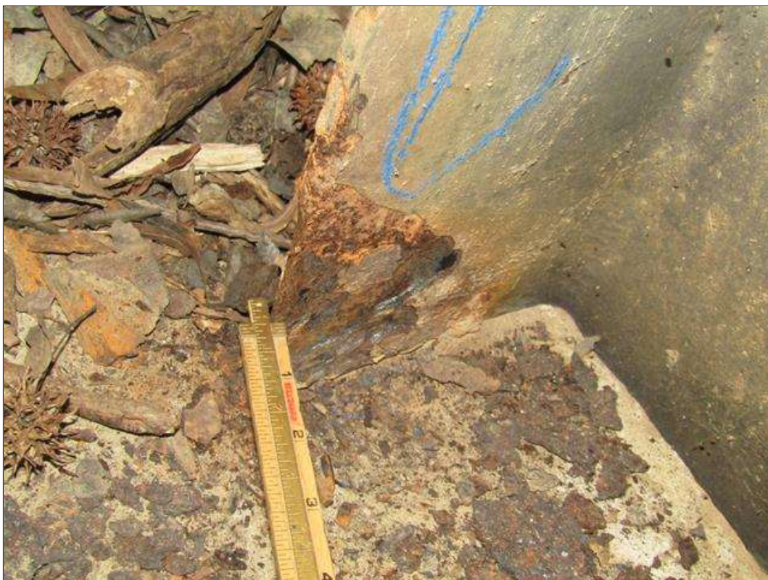
Bent 2 Pile 4: RUST SCALE ON BOTTOM OF NORTH FLANGE ON WEST SIDE UP 4" WITH 1/8" STEEL REMAINING ON 1/2" FLANGE/ PAR
