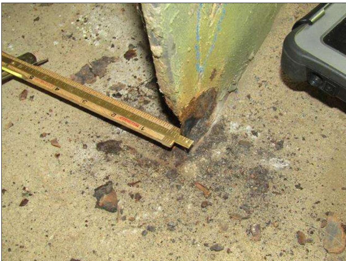
Bent 2 Pile 5: RUST SCALE ON BOTTOM OF SOUTH FLANGE ON WEST SIDE UP 2" X 2" WIDE WITH 1/8" STEEL REMAINING ON 1/2" FLANGE/PAR
