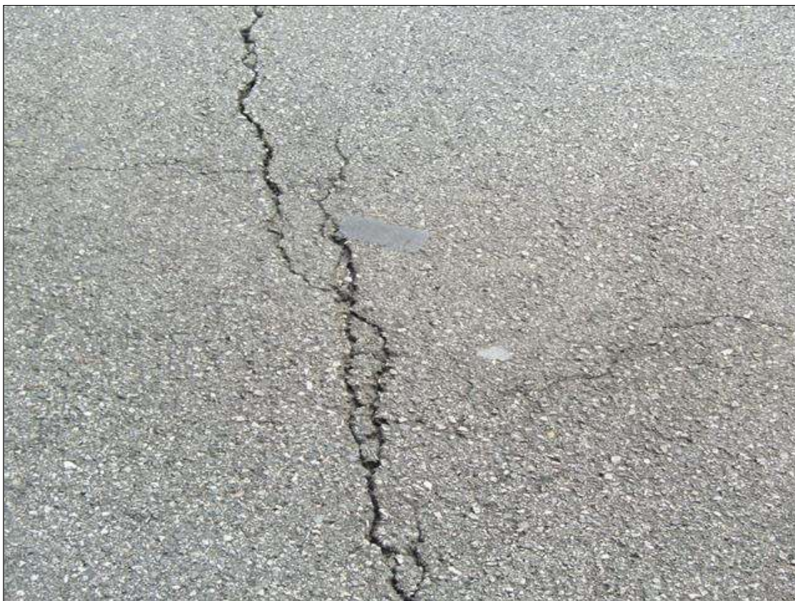
Span 3 Wearing Surface: TRANSVERSE CRACKING OVER END BENT 2 UP TO 1" WIDE
