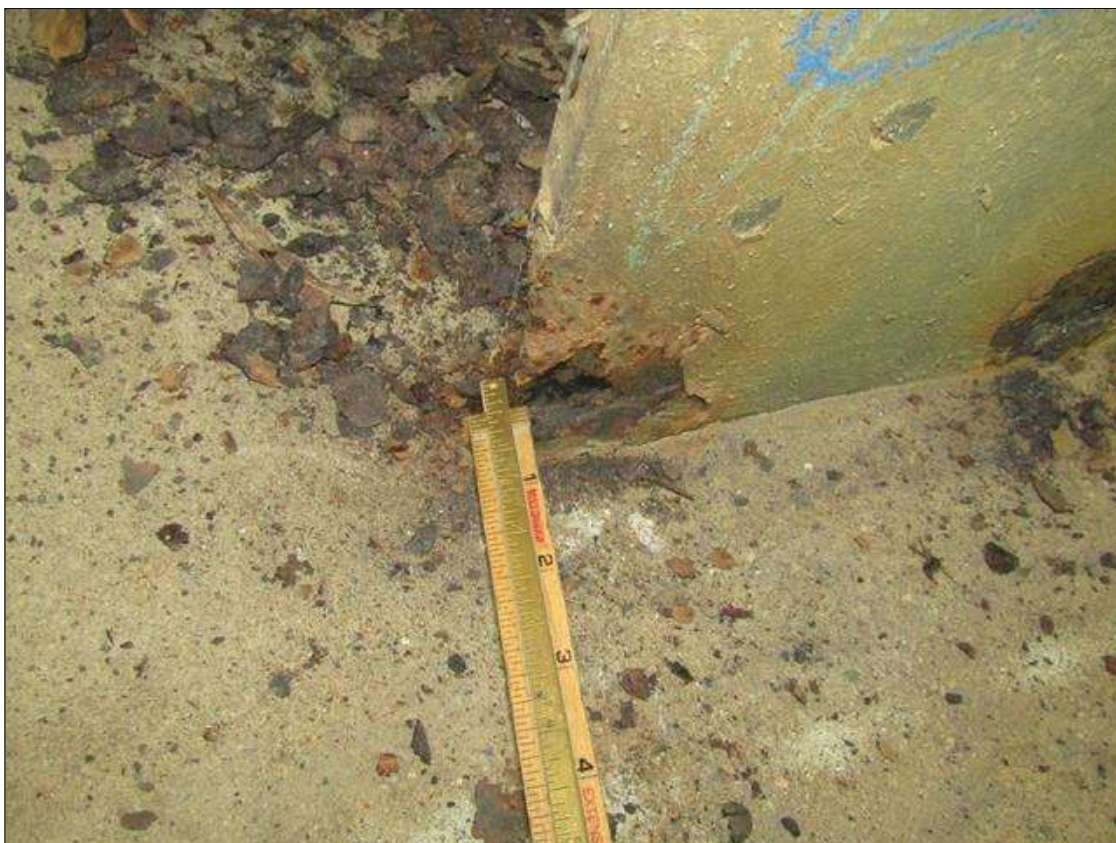
Bent 2 Pile 4: RUST SCALE ON BOTTOM OF SOUTH FLANGE ON WEST SIDE UP 4" X 2" WIDE WITH 1/8" STEEL REMAINING ON 1/2" FLANGE/PAR
