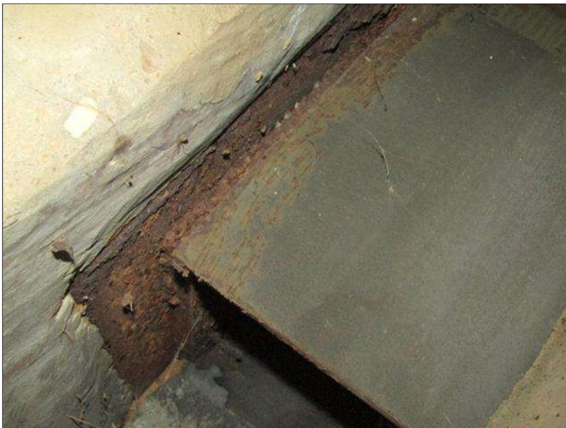
End Bent 2 Pile 2: RUST SCALE ON TOP AT PILE PLATE WITH SURFACE RUST ON TOP OF PILE
