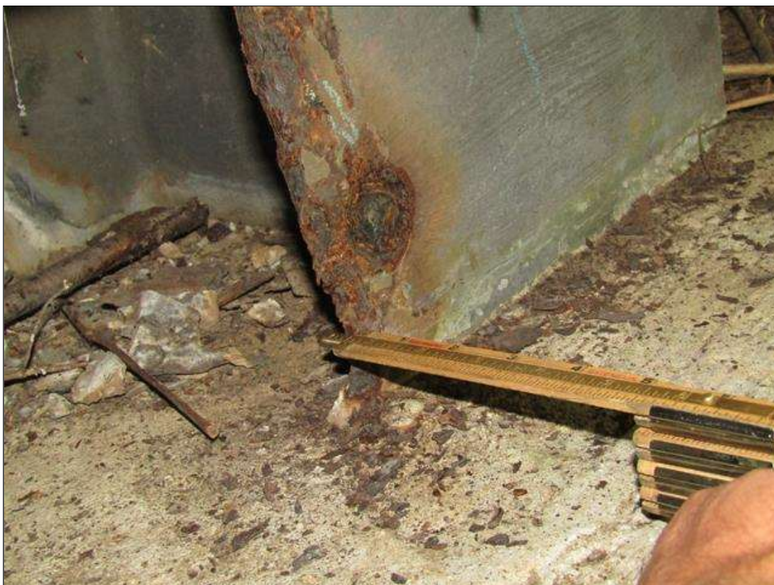
End Bent 1 Pile 1: RUST SCALE WITH STEEL DOWN TO KNIFE EDGE EAST SIDE OF FRONT FLANGE ABOVE FOOTING 46" HIGH x 2" WIDE/ PAR
