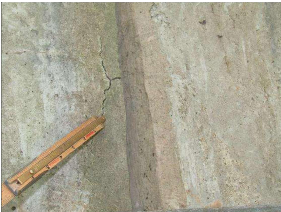
Span 3 Slab 1: CRACK ON END AT PIER 2 UP TO 1/8" WIDE X 6" LONG
