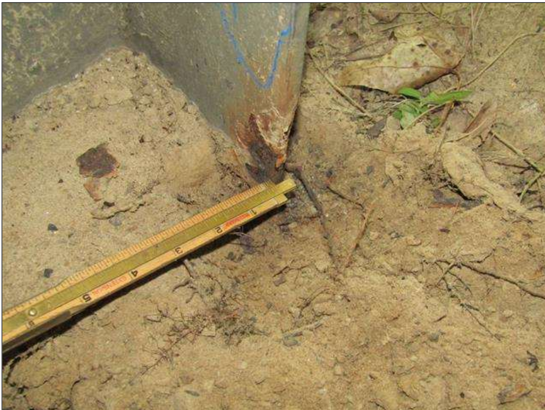
Bent 2 Pile 1: 1/4" STEEL REMAINING ON BOTTOM EAST NORTH FLANGE UP 2" FROM BOTTOM X 2" WIDE/PAR
