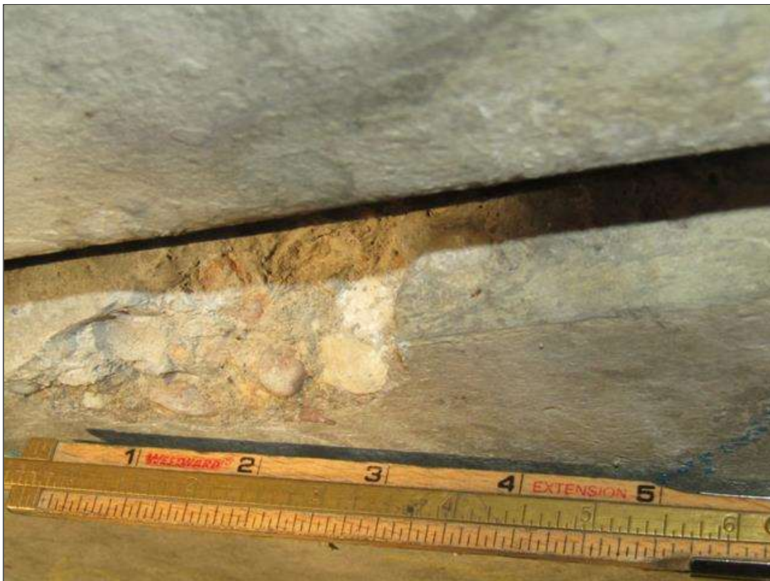
Span 3 Slab 2: TWO CHIP SPALLS ON RIGHT EDGE 5' FROM PIER 2, ONE 4" X 2" X 1/2" DEEP AND OTHER 3" X 2" X 1/2" DEEP
