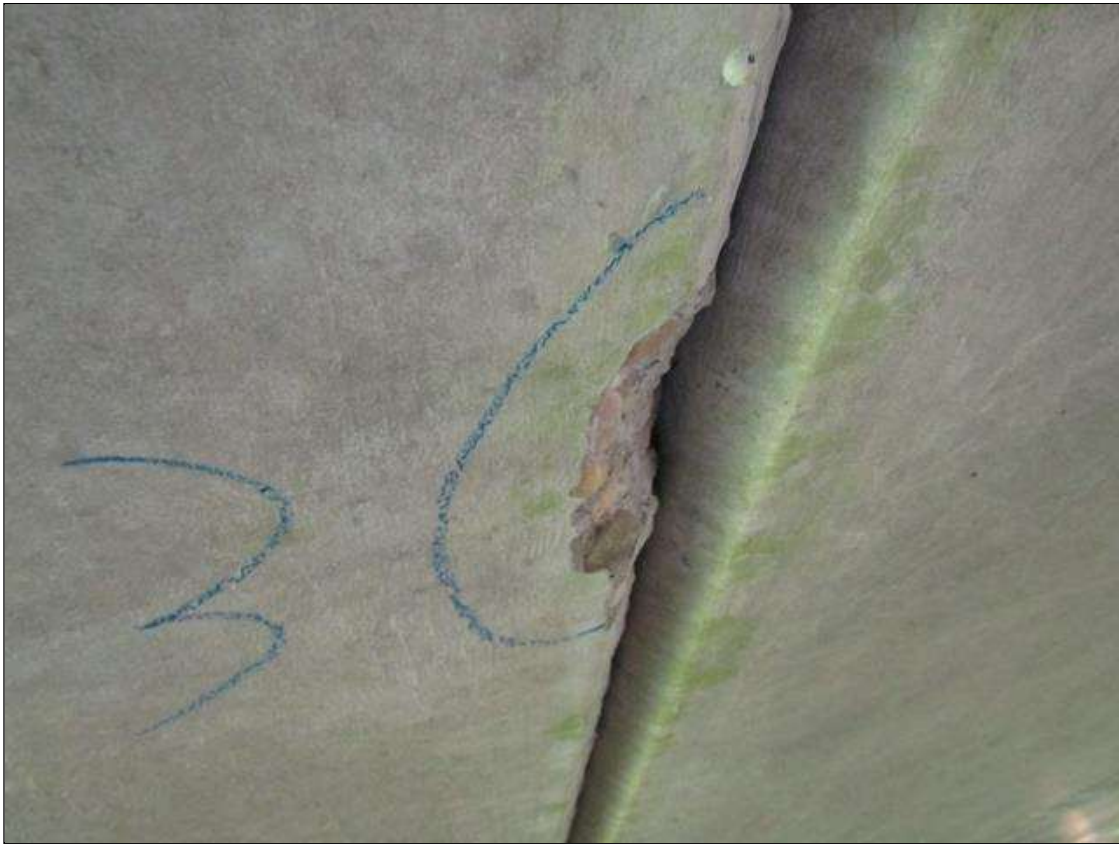
Span 3 Slab 3: SPALL ON RIGHT BOTTOM EDGE 4" LONG X 2" WIDE X 1/4" DEEP 6' FROM PIER 2
