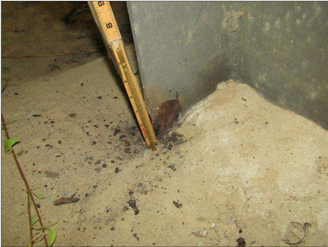
Bent 1 Pile 4: RUST SCALE ON PILE PLATE WITH SURFACE RUST ON TOP AND RUST SCALE ON BOTTOM OF FLANGE ON EAST SIDE ON SOUTH FACE UP 3" X 2" WIDE WITH 1/4" STEEL REMAINING ON 1/2" FLANGE/PAR
