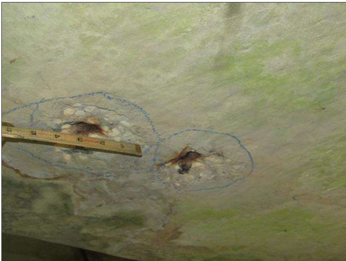
Bent 1 Cap 1: SPALLS ON BOTTOM AT EAST END AND ON BOTTOM BETWEEN PILES 6 -7 UP TO 4" DIAMETER X 1/2" DEEP WITH STEEL EXPOSED
