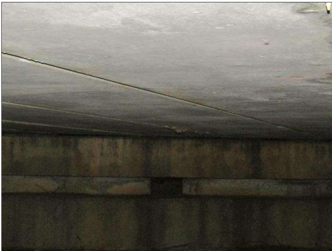
Span 1 Expansion Joint: OLD SEEPAGE STAIN ON END BENT 1 CAP
