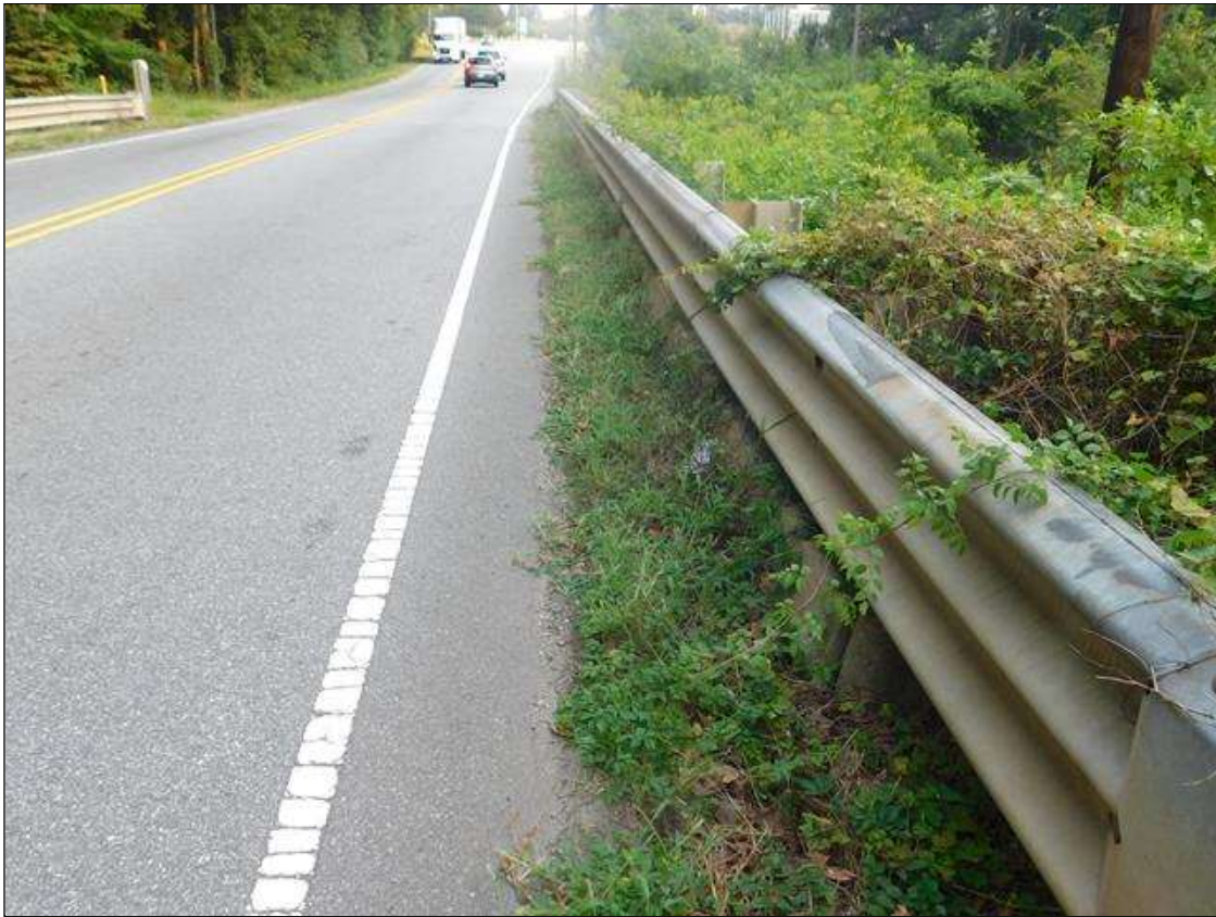
DEBRIS AND VEGETATION GROWING ALONG RAILS
