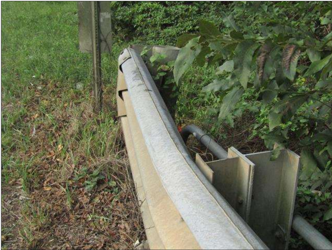
Span 1 Left Bridge Rail: RAIL BENT AT POST 1 GOING TO SOUTH END
