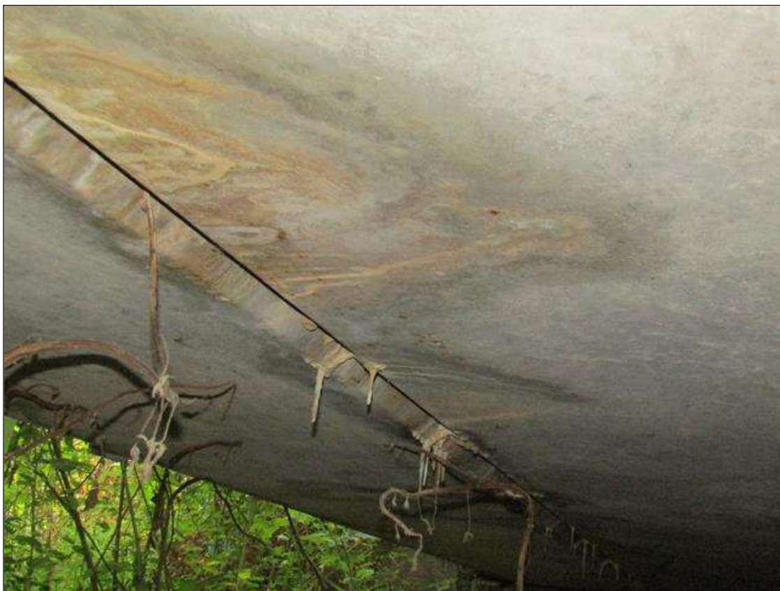
Span 1 Slab 11: EFFLO BUILT UP AND STAIN ON BOTTOM FROM BETWEEN SLABS
