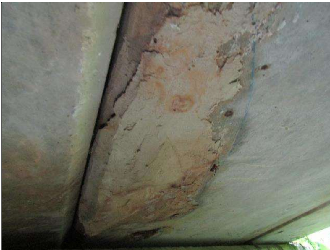
Span 1 Slab 11: PATCH AREA CRACKING ON BOTTOM NEAR PIER
