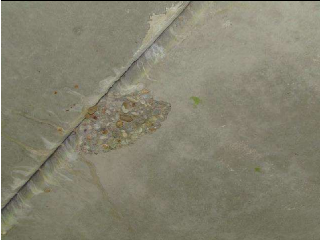
Span 2 Slab 5: SPALL ON LEFT BOTTOM CORNER MID SPAN 10" LONG X 5" WIDE X 1" DEEP
