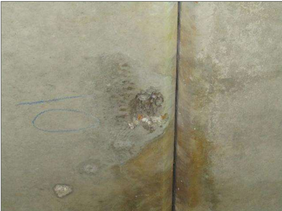
Span 2 Slab 10: 4" X 2" HONEYCOMB AREA ON BOTTOM NEAR PIER 2
