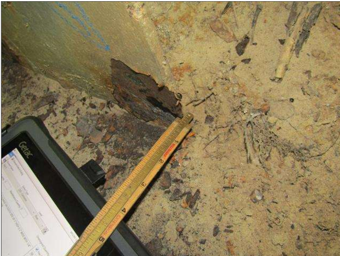
Bent 2 Pile 3: RUST SCALE ON BOTTOM EAST FLANGE ON SOUTH SIDE UP 3" HIGH X 2" WIDE WITH 1/4" STEEL REMAINING ON 1/2" FLANGE/PAR
