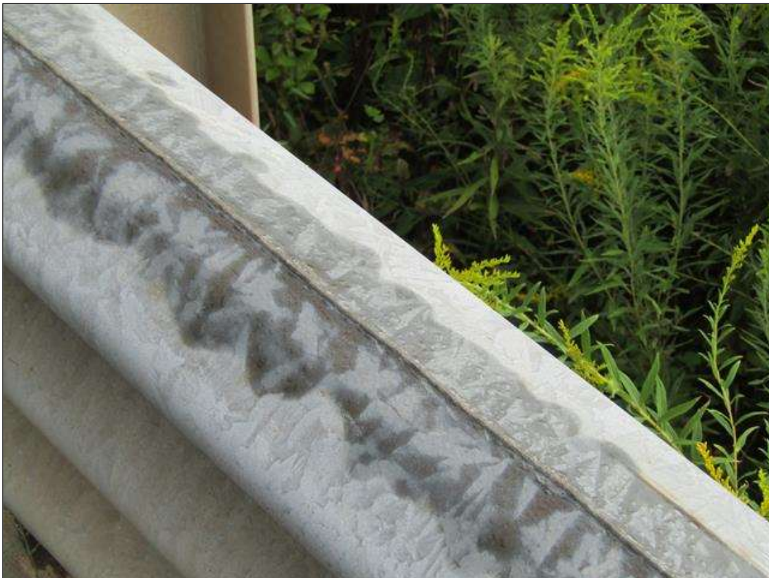
Span 3 Right Bridge Rail - Protective System: SUBSTANTIALLY EFFECTIVE ON TOP
