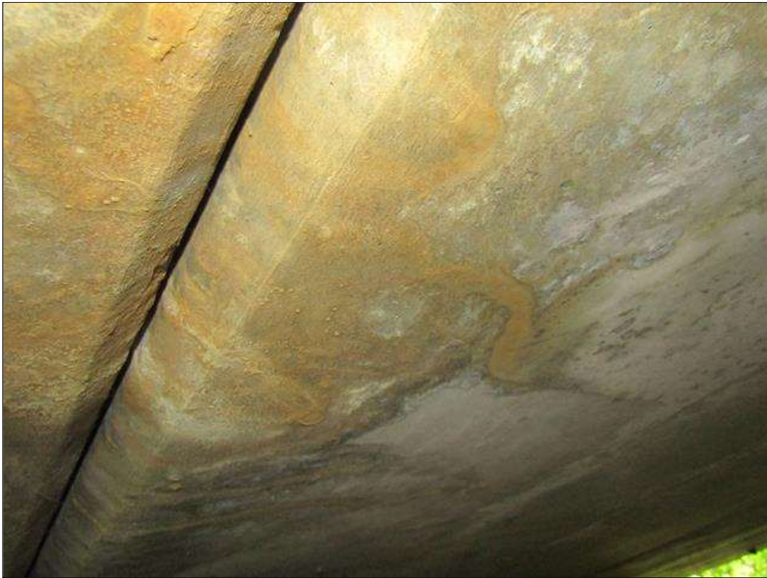
Span 1 Slab 4: EFFLO AND STAIN ON BOTTOM FROM BETWEEN SLABS
