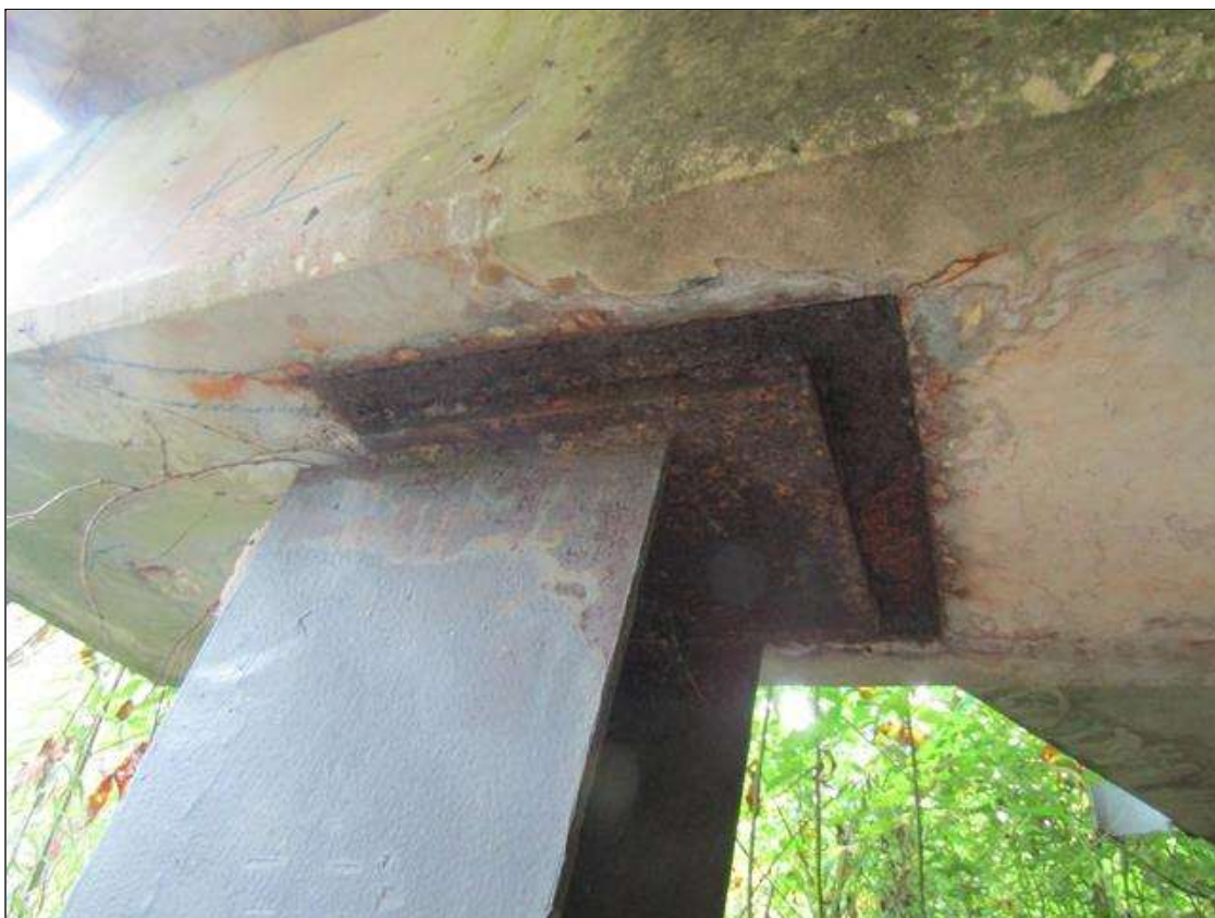
Bent 1 Pile 7: RUST SCALE ON PILE PLATE WITH SURFACE RUST ON TOP OF PILE
