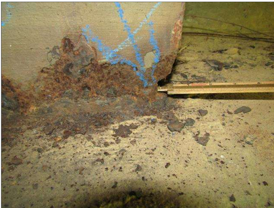
End Bent 2 Pile 5: RUST SCALE ON BOTTOM FRONT FLANGE ON ACROSS WIDTH WITH 1/4" SECTION LOSS AND COMPLETE SECTION LOSS ON BOTTOM EAST SIDE 2" X 1" AREA ON 1/2" FLANGE/PAR
