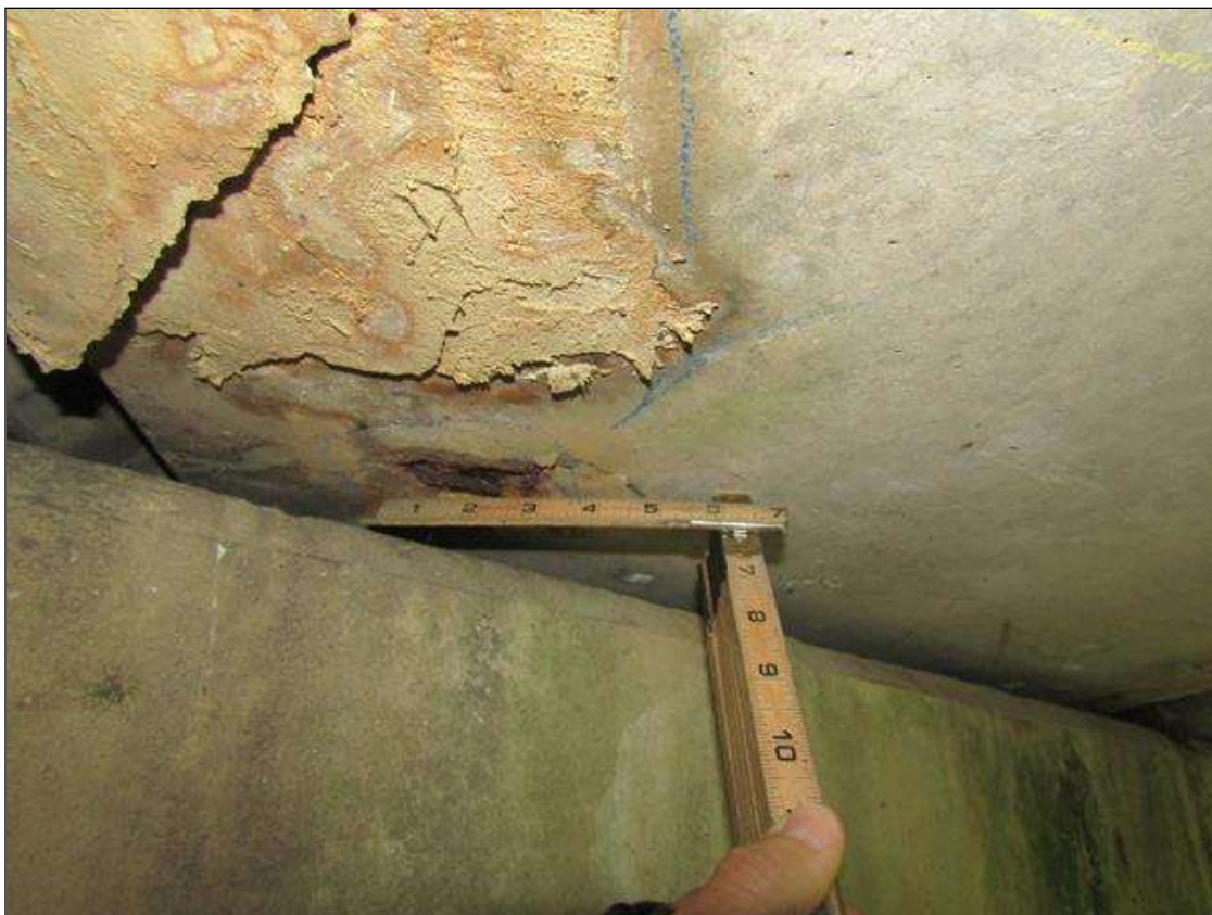
Span 1 Slab 11: POPOUT SPALL ON BOTTOM AT PIER 3" DIAMETER X 1/4" DEEP STEEL TO CLOSE TO SURFACE
