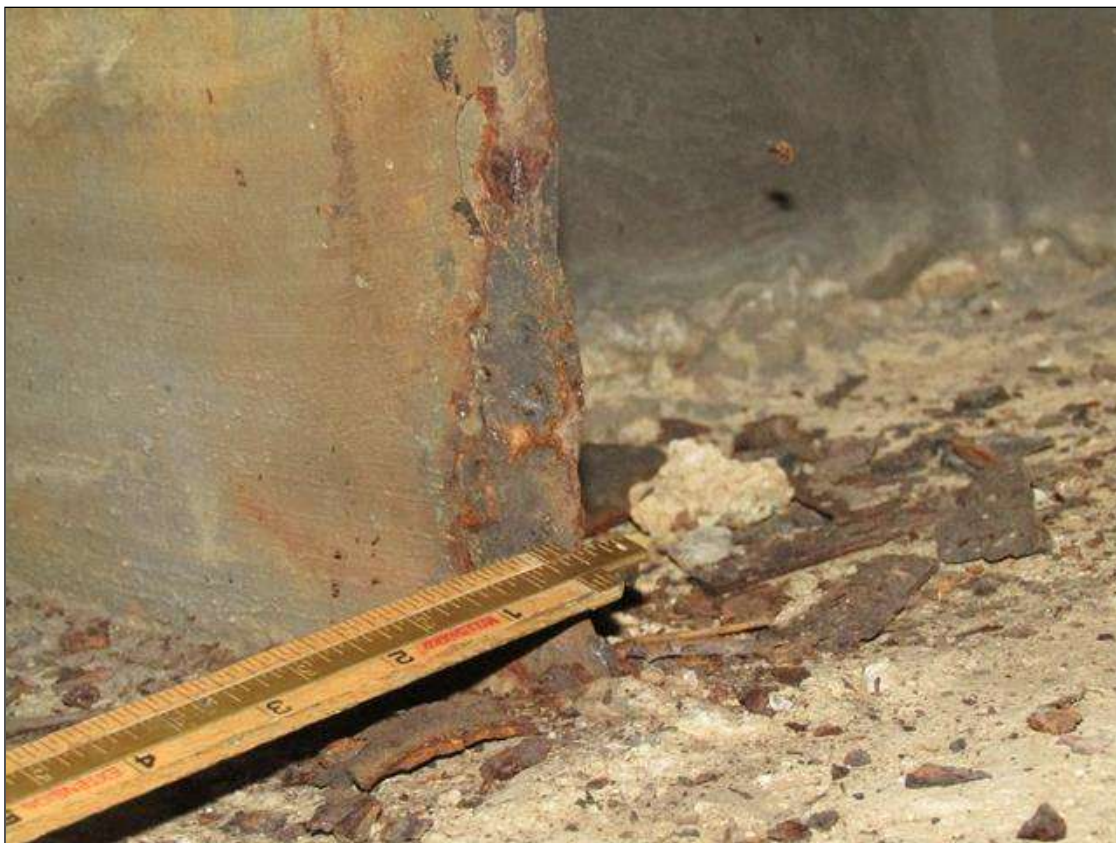
End Bent 1 Pile 2: 1/4" STEEL REMAINING ON FRONT WEST EDGE 3" HIGH X 1" WIDE/PAR
