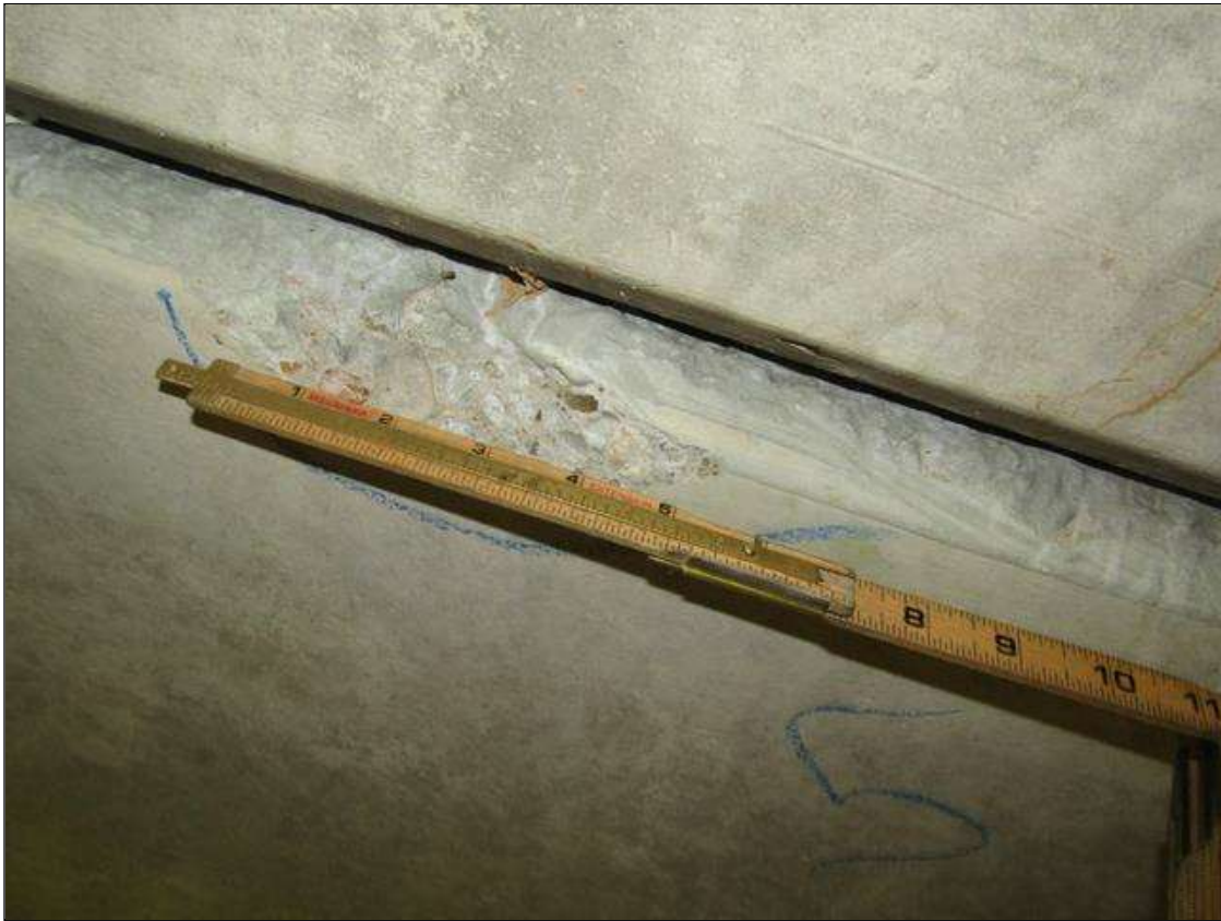
Span 3 Slab 5: SPALL ON RIGHT BOTTOM EDGE 5" LONG X 2" WIDE X 1/2" DEEP NEAR MID SPAN
