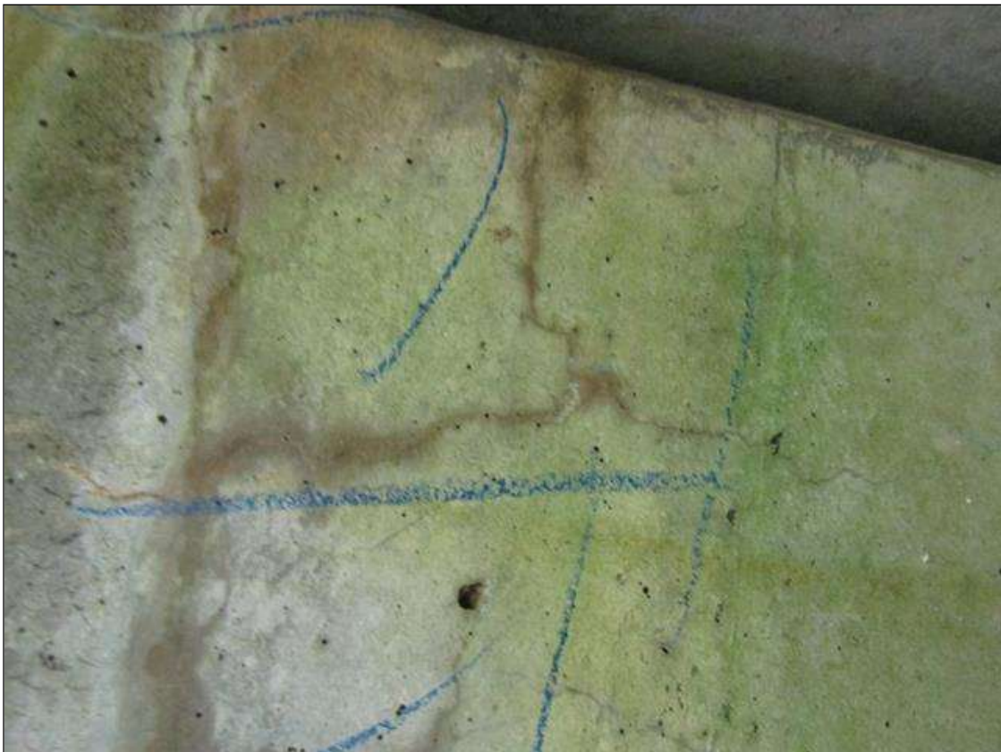
End Bent 2 Cap 1: HAIRLINE LONGITUDINAL AND MAP CRACKING ON ENDS
