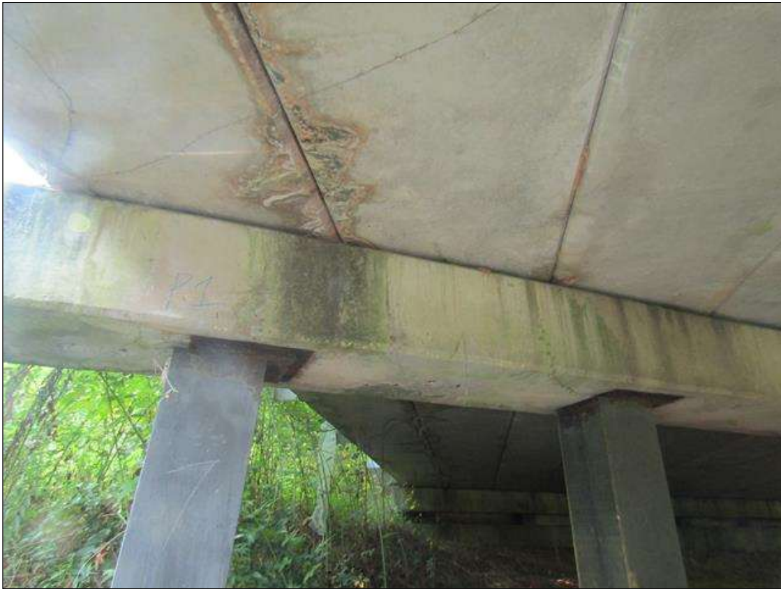
Span 2 Expansion Joint: OLD MOISTURE STAIN ON PIER 1 CAP
