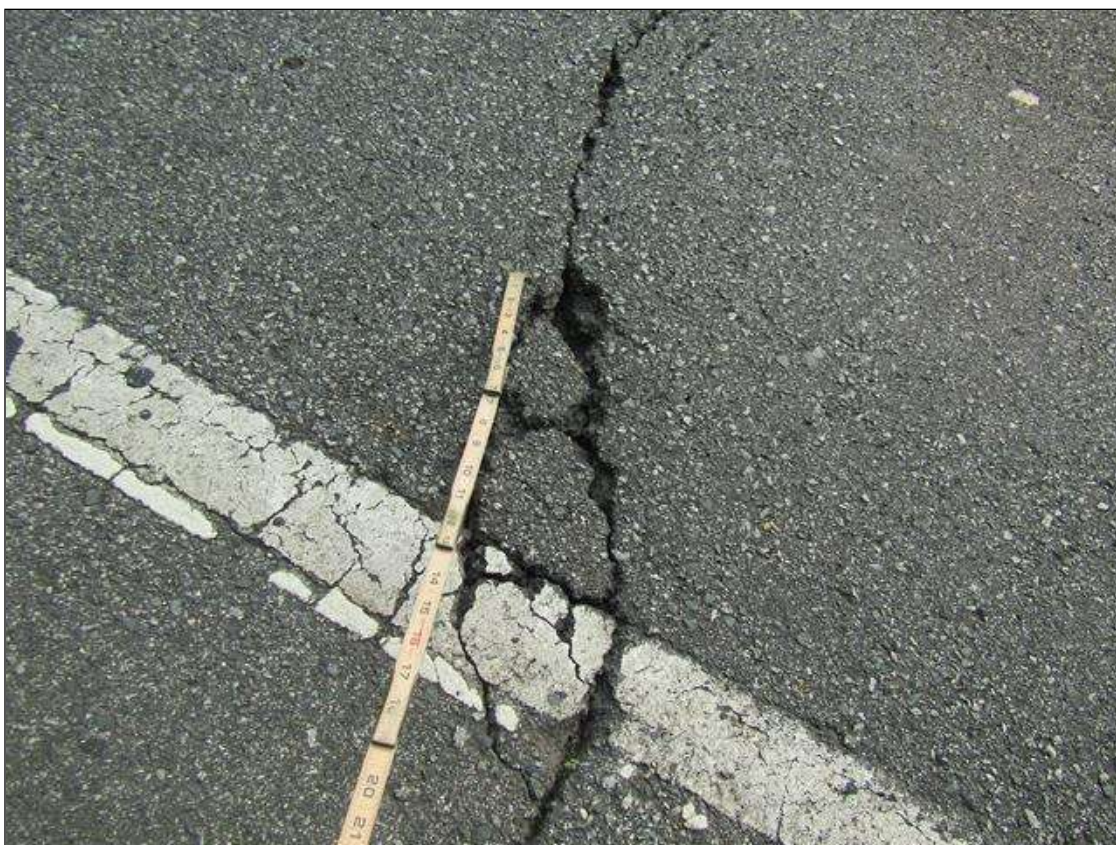
Span 3 Wearing Surface: ASPHALT BUSTING UP OVER END BENT 2 IN SBL NEAR WHITE LINE 18" x 5"
