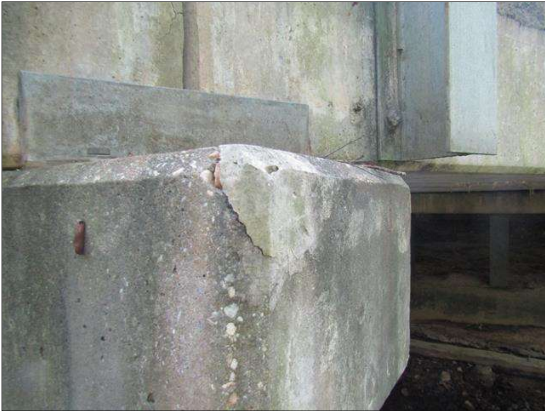
Bent 2 Cap 1: PATCH HAS CRACK ON TOP AT NORTHWEST CORNER
