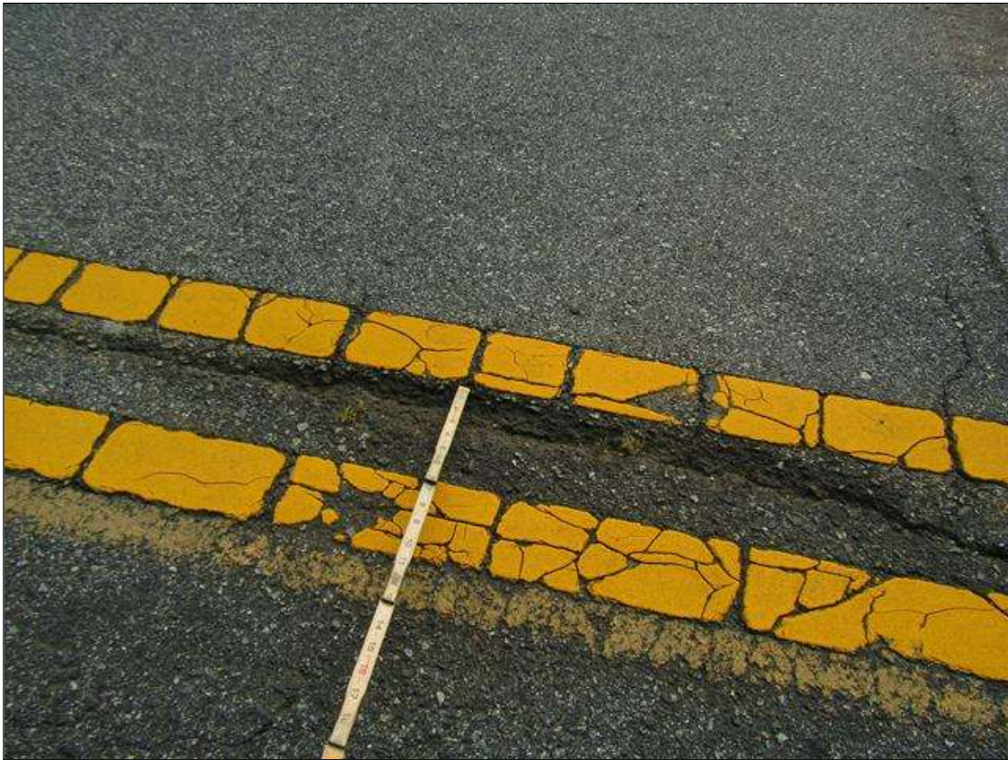
Span 3 Wearing Surface: ASPHALT SEPARATED IN CENTER NEAR END BENT 2 x 4" WIDE
