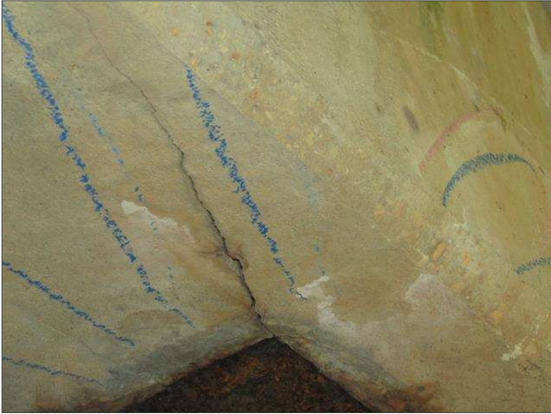
Bent 2 Cap 1: CRACKING ON BOTTOM AROUND CORNERS OF PILE PLATES 1/64" WIDE UP TO 8" LONG
