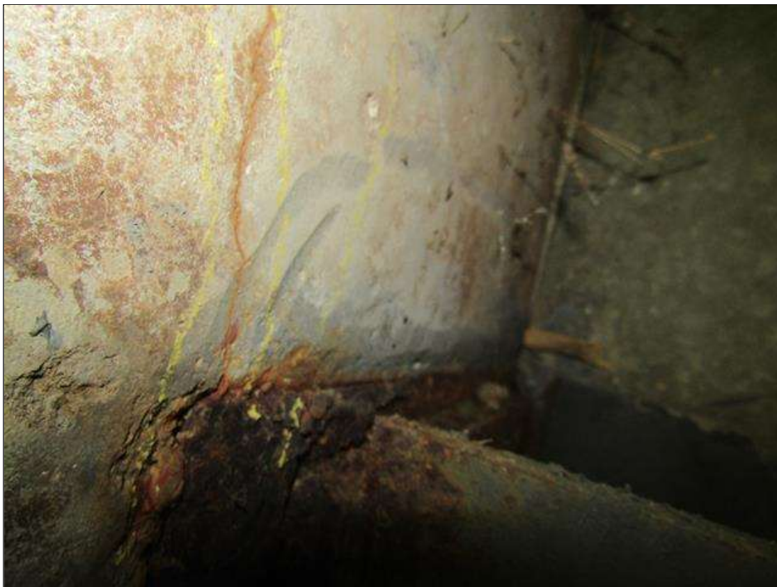
End Bent 2 Cap 1: CRACKING ON BOTTOM AROUND CORNERS OF PILES 1/64" WIDE UP TO 6" LONG
