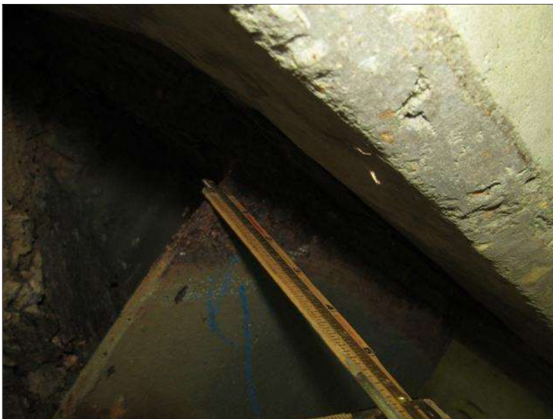
End Bent 2 Pile 1: RUST SCALE ON TOP OF SOUTH FLANGE ON WEST END 3" LONG X 2" WIDE WITH 1/4" STEEL REMAINING ON 1/2" FLANGE/PAR
