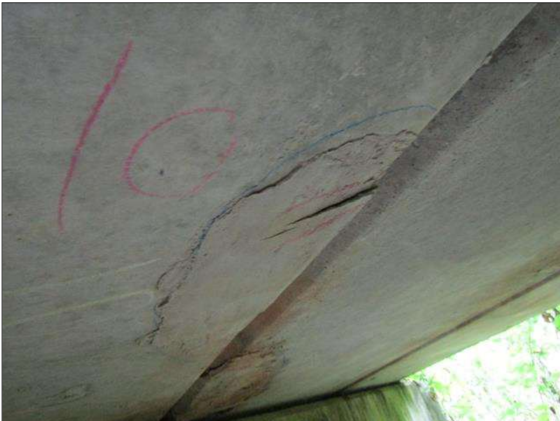
Span 1 Slab 10: PATCH AREA HAS CRACK ON BOTTOM NEAR PIER
