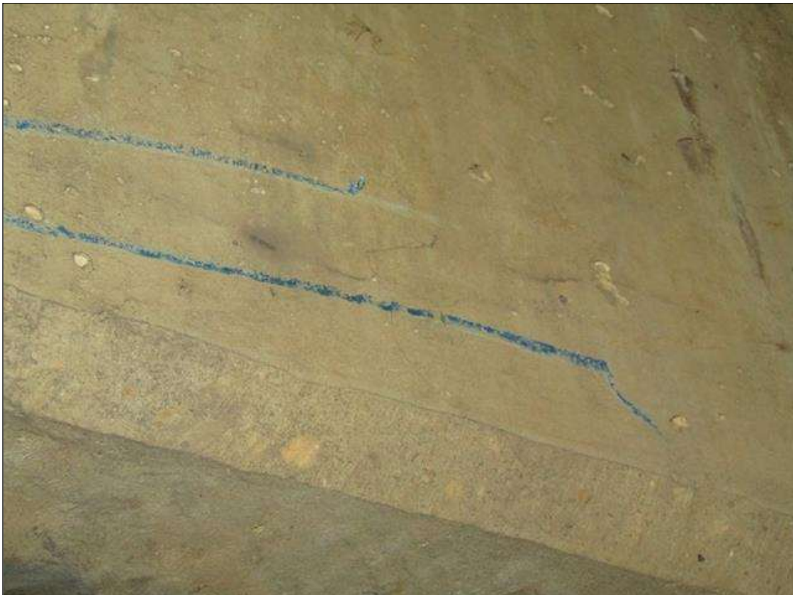
Bent 1 Cap 1: HAIRLINE LONGITUDINAL CRACKS ON BOTH FACES OVER PILES
