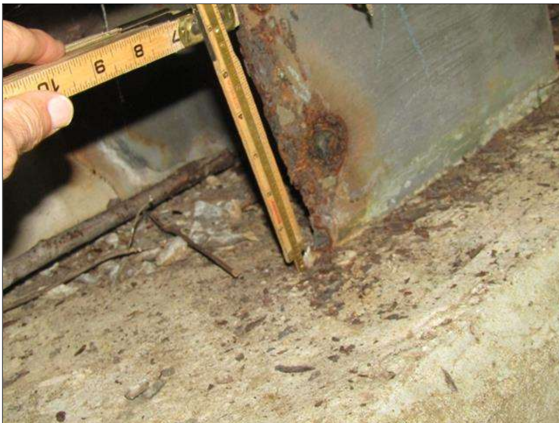
End Bent 1 Pile 1: RUST SCALE WITH STEEL DOWN TO KNIFE EDGE EAST SIDE OF FRONT FLANGE ABOVE FOOTING 46" HIGH x 2" WIDE/ PAR
