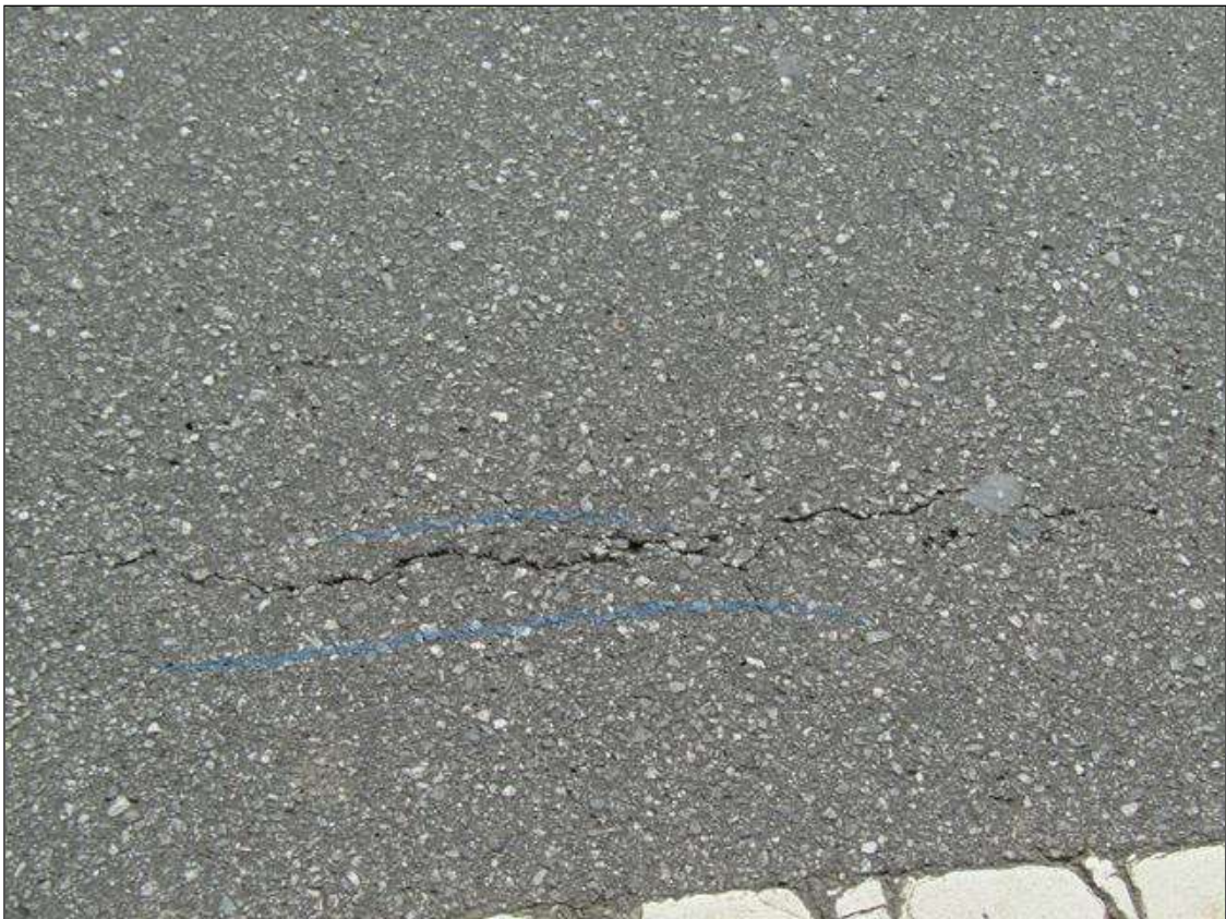
Span 2 Wearing Surface: LONGITUDINAL CRACK 1/16" WIDE IN SBL
