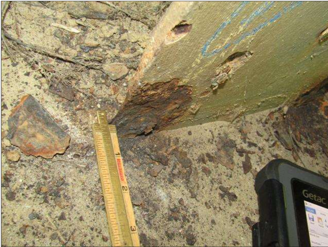
Bent 2 Pile 3: RUST SCALE ON BOTTOM WEST FLANGE ON SOUTH SIDE UP 3" HIGH X 2" WIDE WITH 1/8" STEEL REMAINING ON 1/2" FLANGE/PAR
