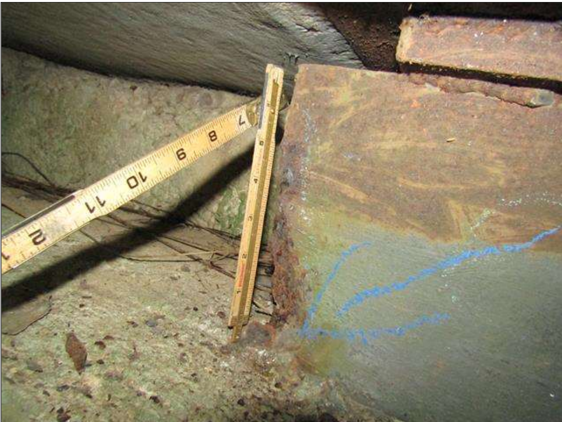
End Bent 1 Pile 6: RUST SCALE WITH REMAINING STEEL DOWN TO KNIFE EDGE ON EAST SIDE FRONT FLANGE UP 5" HIGH ABOVE FOOTING X 2" WIDE WITH EDGE BREAKING OFF/ PAR
