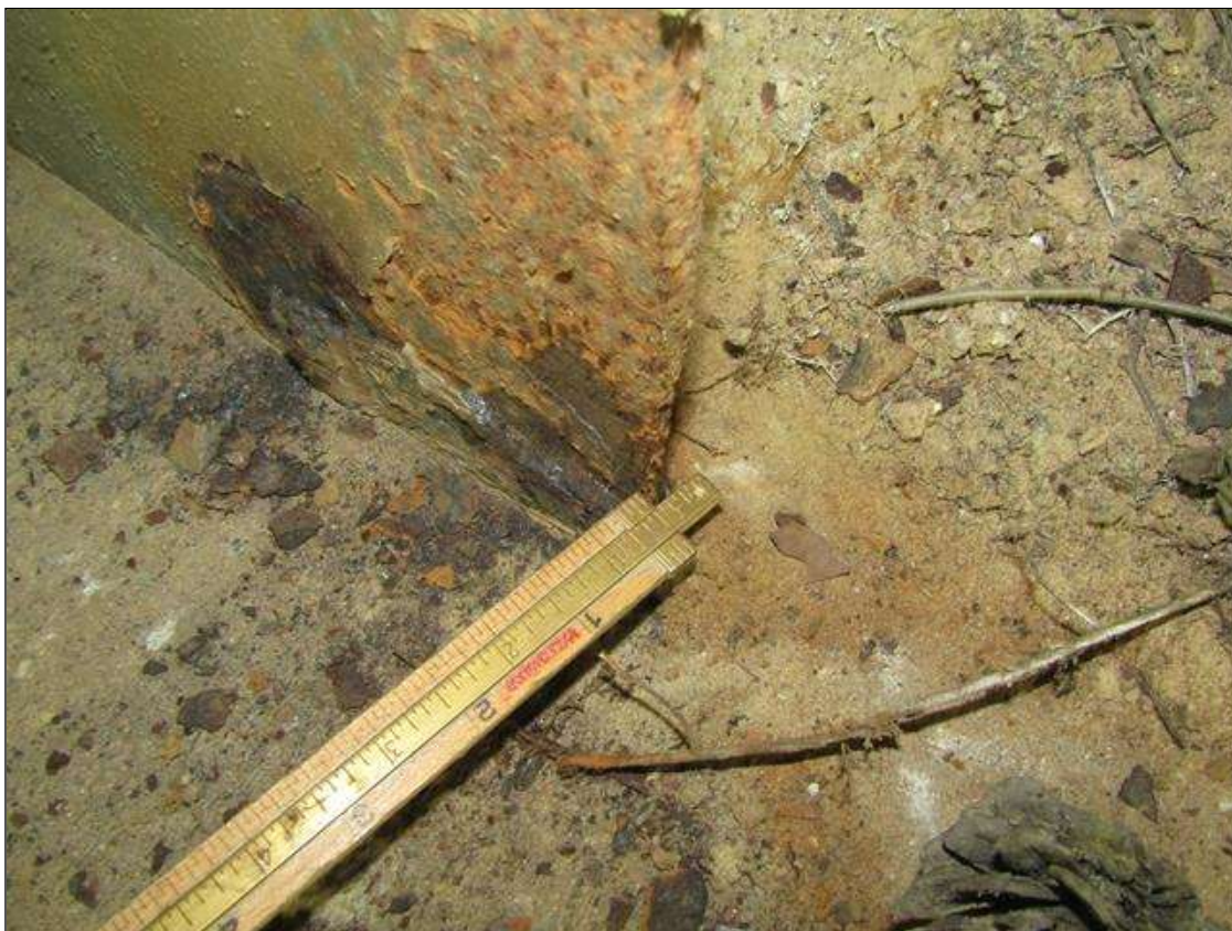
Bent 2 Pile 4: RUST SCALE ON BOTTOM OF SOUTH FLANGE ON EAST SIDE UP 4" WITH 1/8" STEEL REMAINING ON 1/2" FLANGE/PAR
