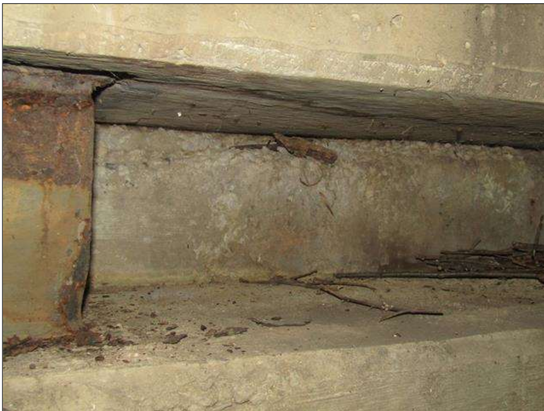
End Bent 1 Abutment: CONCRETE VOIDS IN TOP WHERE CONCRETE WAS POURED BETWEEN PILES 1-4
