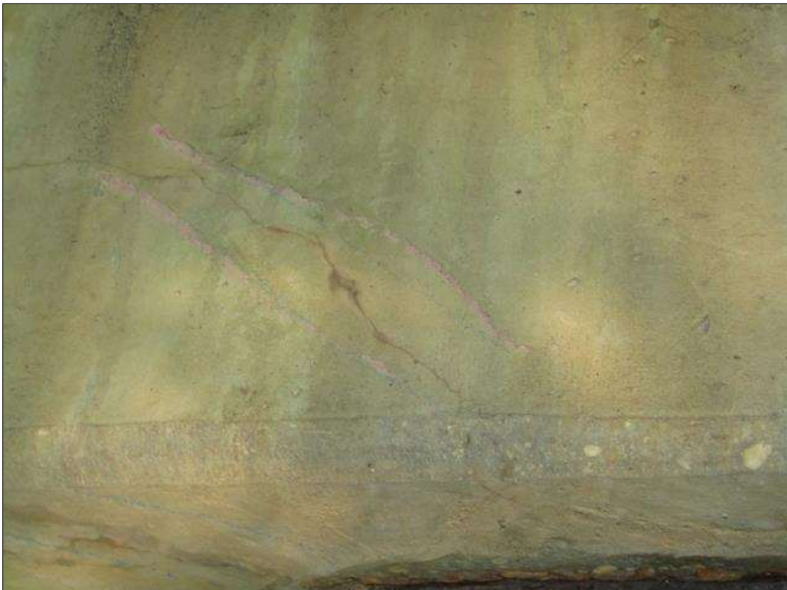
Bent 2 Cap 1: HAIRLINE DIAGONAL ON SOUTH FACE OVER PILE 2
