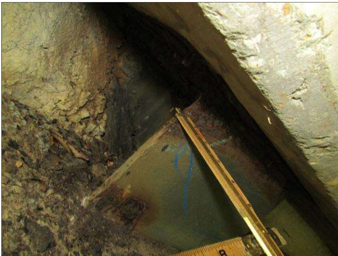
End Bent 2 Pile 1: RUST SCALE ON TOP OF SOUTH FLANGE ON WEST END 3" LONG X 2" WIDE WITH 1/4" STEEL REMAINING ON 1/2" FLANGE/PAR
