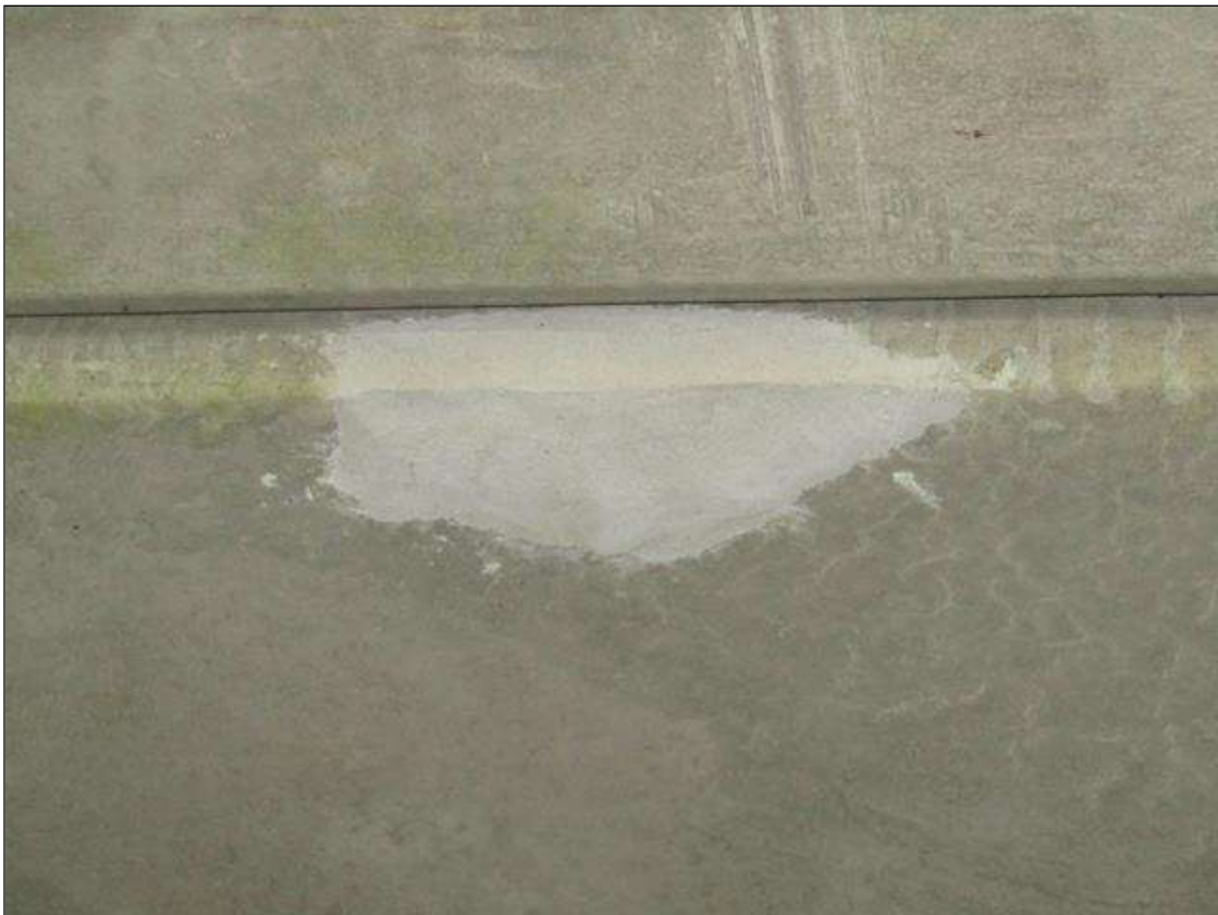
Span 2 Slab 4: PATCH AREA ON BOTTOM AT MID SPAN AND NEAR PIER 1
