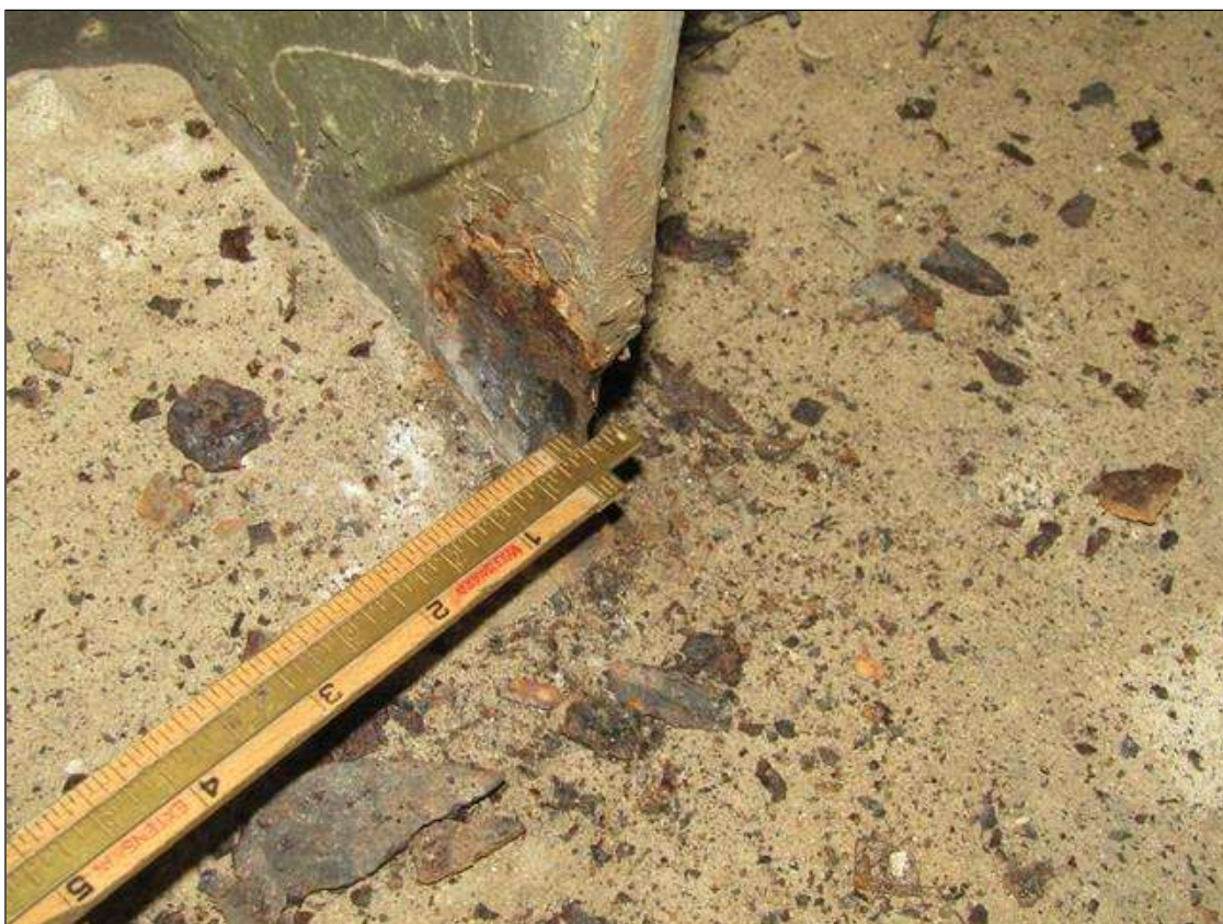
Bent 1 Pile 3: 1/8" STEEL REMAINING ON BACK EAST FLANGE AT BOTTOM UP 3"/PAR
