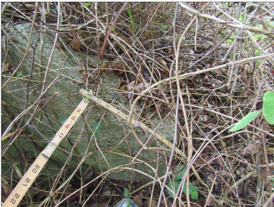
End Bent 1 Abutment: SPALL AT SOUTHWEST CORNER 12" LONG X 4" WIDE X 1" DEEP
