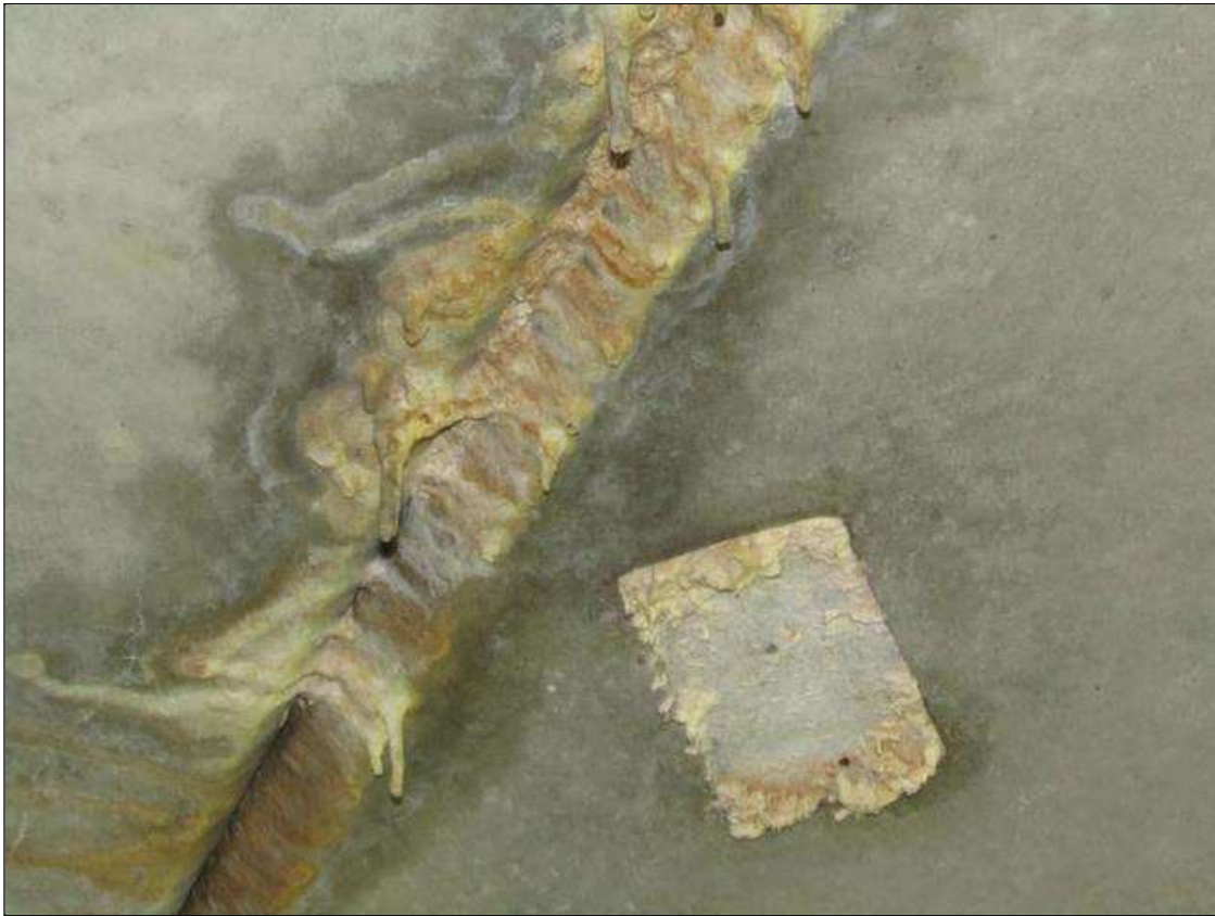
Span 2 Slab 1: EFFLO BUILT UP WITH STAIN ON BOTTOM FROM BETWEEN SLABS
