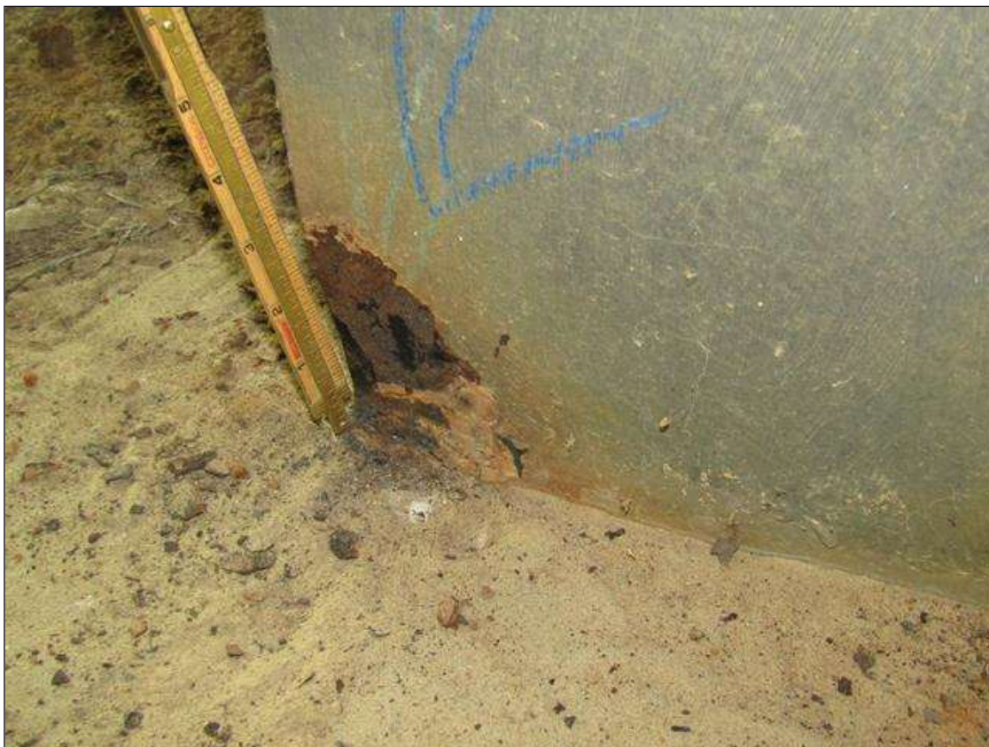
Bent 2 Pile 2: RUST SCALE ON BOTTOM WEST FLANGE ON SOUTH SIDE UP 3" HIGH X 2" WIDE WITH 1/8" STEEL REMAINING ON 1/2" FLANGE/PAR
