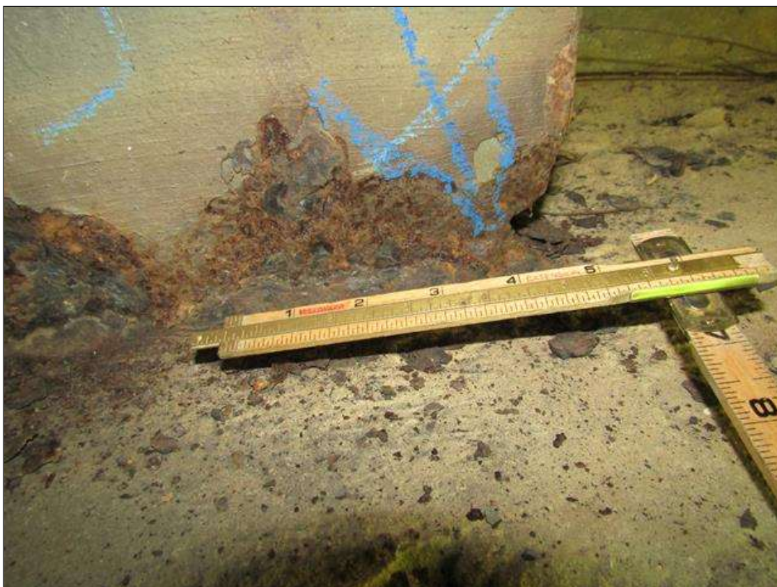
End Bent 2 Pile 5: RUST SCALE ON BOTTOM FRONT FLANGE ON ACROSS WIDTH WITH 1/4" SECTION LOSS AND COMPLETE SECTION LOSS ON BOTTOM EAST SIDE 2" X 1" AREA ON 1/2" FLANGE/PAR
