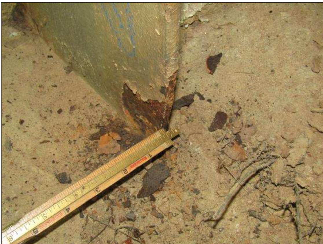
Bent 2 Pile 2: RUST SCALE ON BOTTOM EAST FLANGE ON SOUTH SIDE UP 3" HIGH X 2" WIDE WITH 1/8" STEEL REMAINING ON 1/2" FLANGE/PAR
