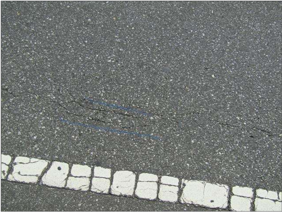
Span 1 Wearing Surface: LONGITUDINAL CRACK 1/16" WIDE IN SBL
