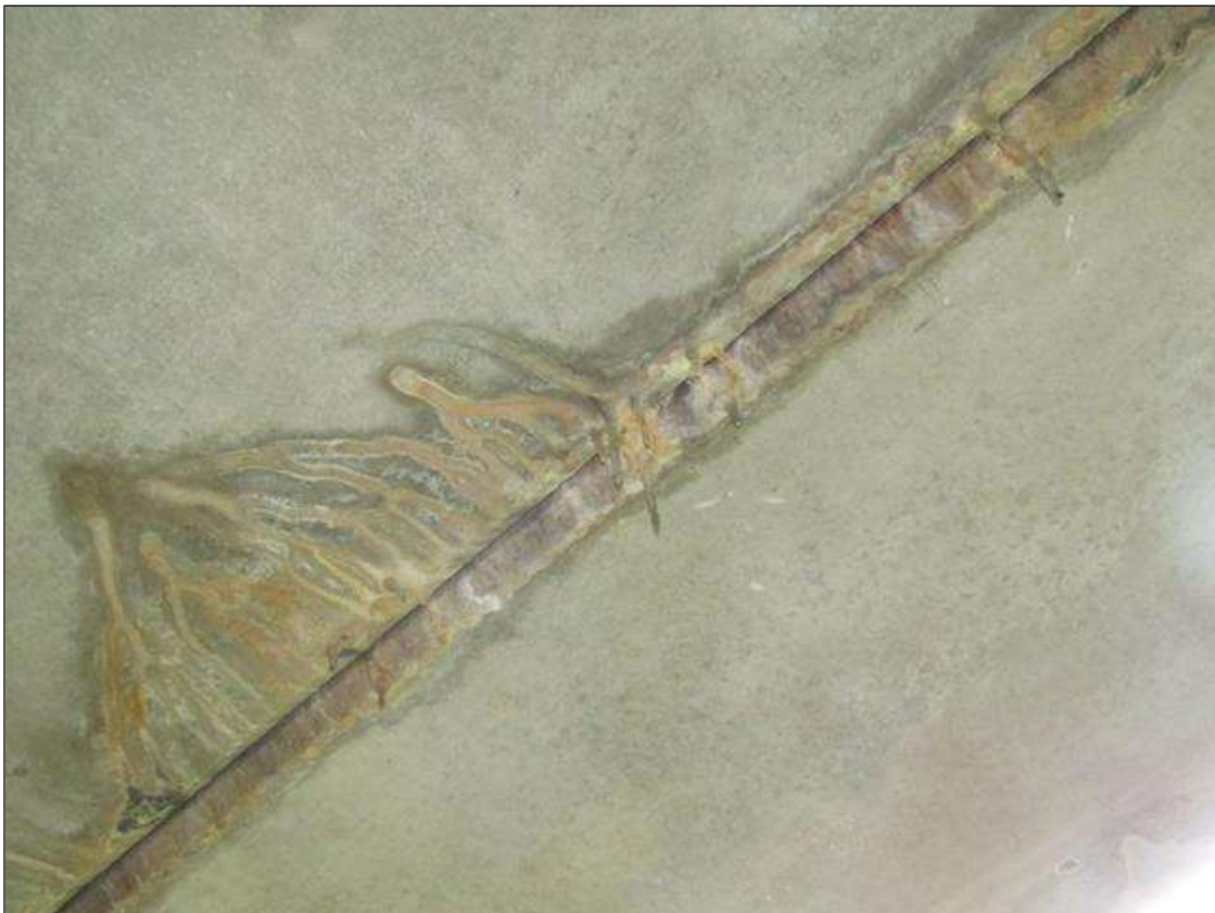
Span 2 Slab 12: EFFLO BUILT UP ON BOTTOM FROM BETWEEN SLABS
