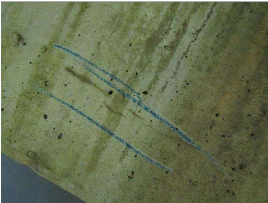
Bent 2 Cap 1: HAIRLINE LONGITUDINAL CRACK ON BOTH FACES ON EAST END AND OVER PILE 3
