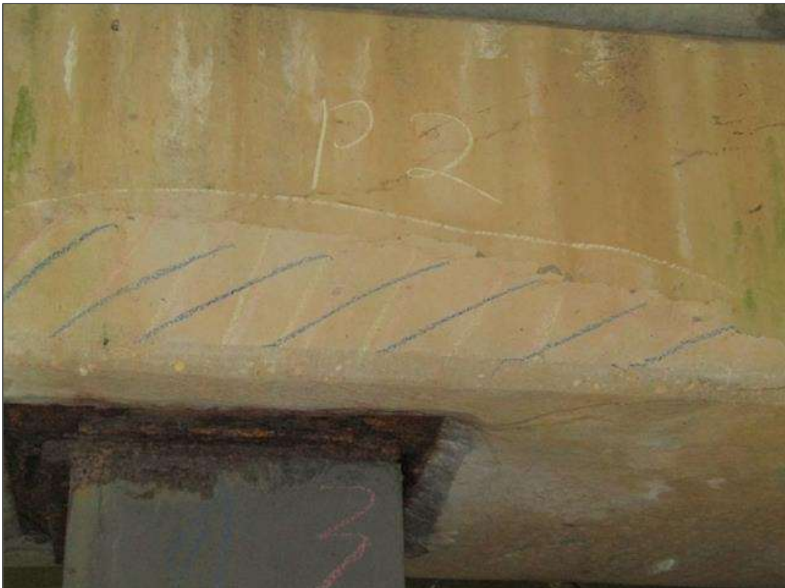
Bent 2 Cap 1: DELAM AREA 3' LONG X 5" WIDE OVER PILE 3 ON SOUTH FACE
