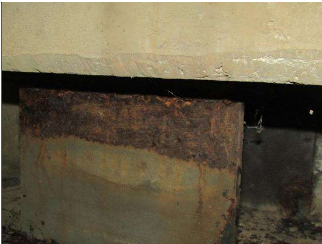
End Bent 1 Pile 2: SURFACE RUST ON PLATE AND TOP OF PILE
