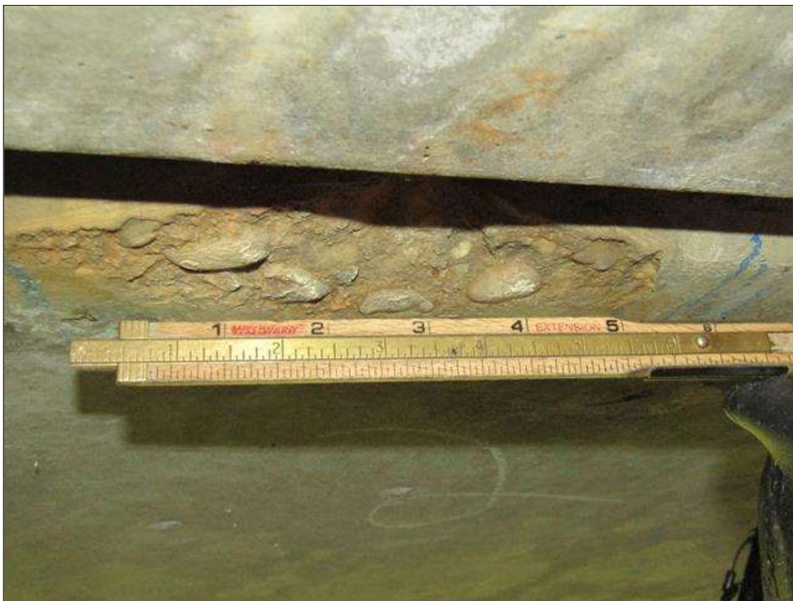
Span 3 Slab 2: TWO CHIP SPALLS ON RIGHT EDGE 5' FROM PIER 2, ONE 4" X 2" X 1/2" DEEP AND OTHER 3" X 2" X 1/2" DEEP
