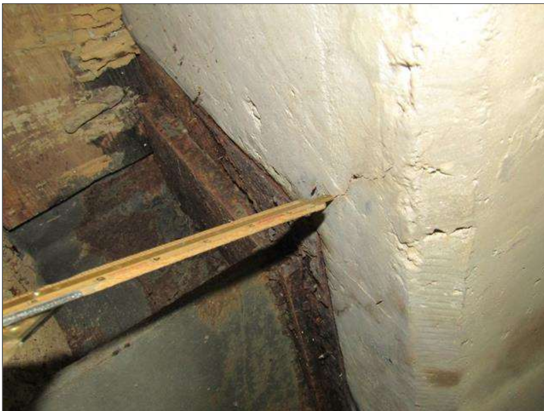
End Bent 1 Cap 1: CRACKING ON BOTTOM AROUND CORNERS OF PILES 1/64" WIDE UP TO 6" LONG
