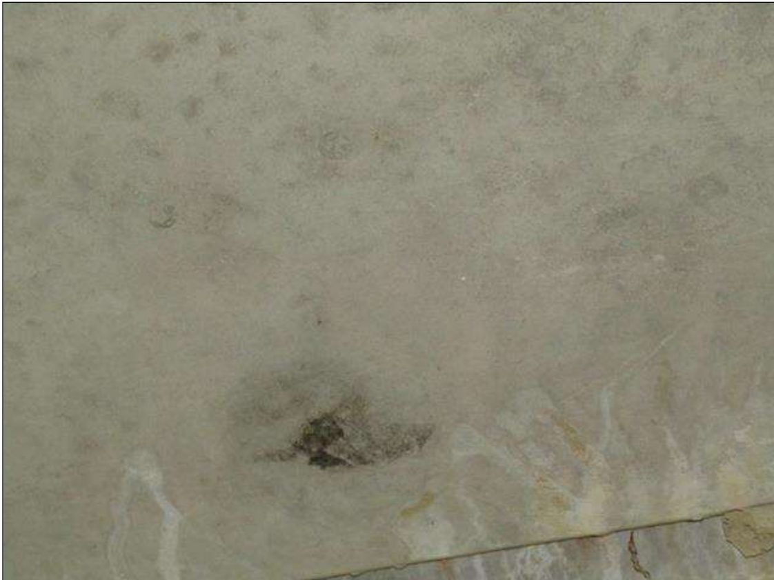
Span 2 Slab 7: 2" HONEYCOMB AREA ON BOTTOM MID SPAN
