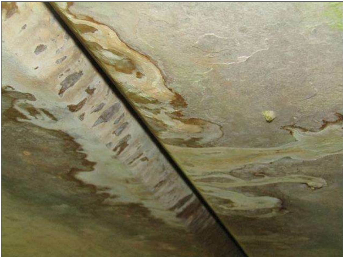
Span 3 Slab 2: EFFLO ON BOTTOM FROM BETWEEN SLABS
