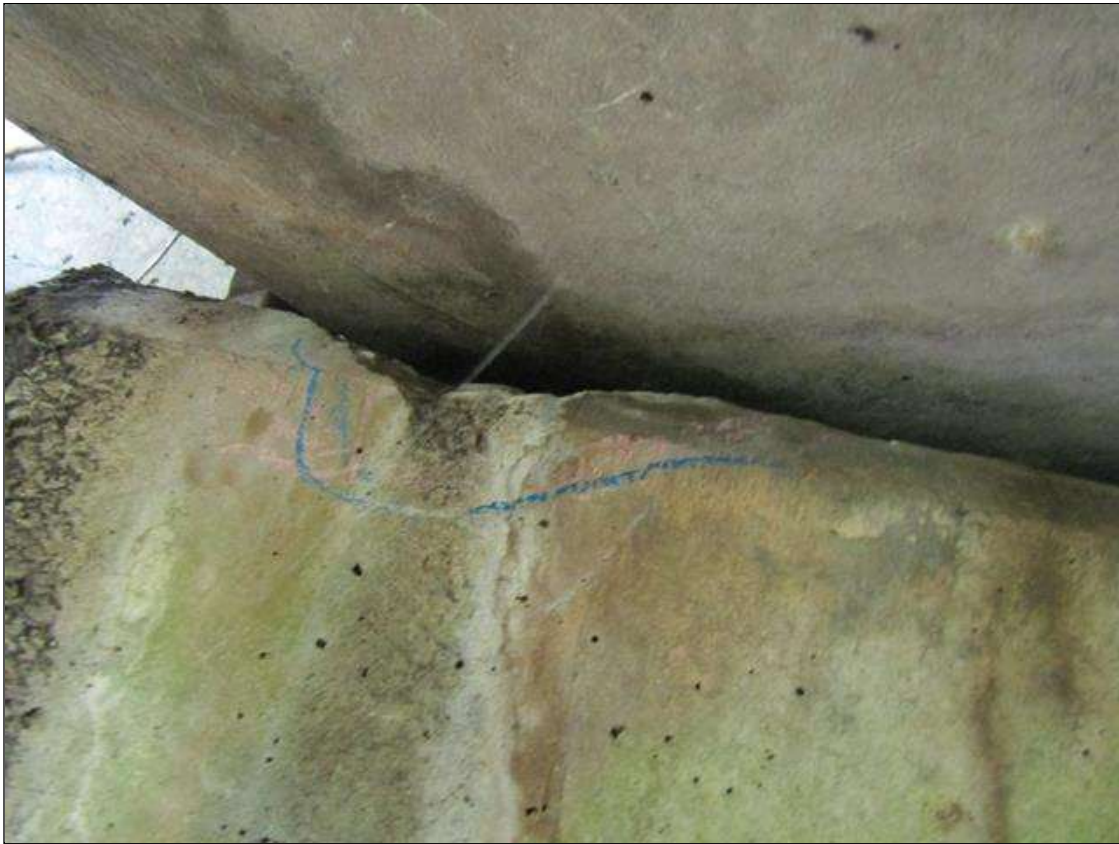
End Bent 2 Cap 1: SPALL ON TOP UNDER SLAB 1, 4" X 2" X 1/2" DEEP
