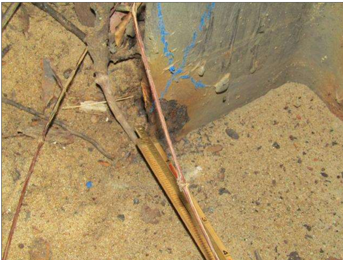
Bent 2 Pile 6: RUST SCALE ON BOTTOM OF SOUTH FLANGE ON EAST SIDE UP 3" X 2" WIDE WITH 1/8" STEEL REMAINING ON 1/2" FLANGE/PAR
