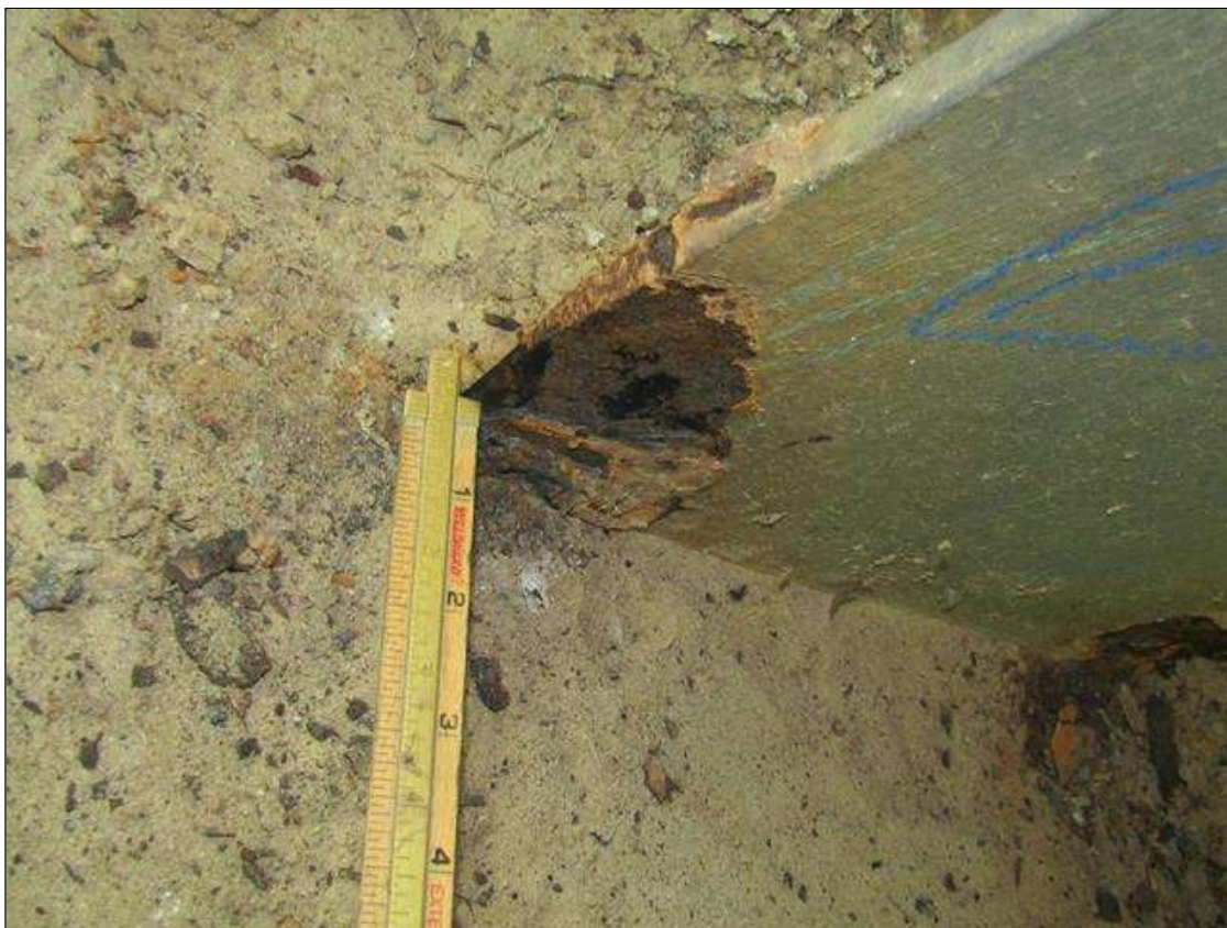
Bent 2 Pile 2: RUST SCALE ON BOTTOM WEST FLANGE ON SOUTH SIDE UP 3" HIGH X 2" WIDE WITH 1/8" STEEL REMAINING ON 1/2" FLANGE/PAR
