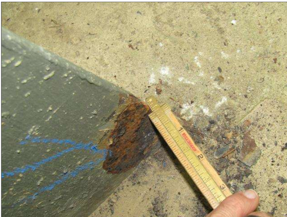
Bent 1 Pile 1: 1/4" STEEL REMAINING ON BOTTOM WEST SPAN 2 FLANGE UP 3" x 2" WIDE/PAR
