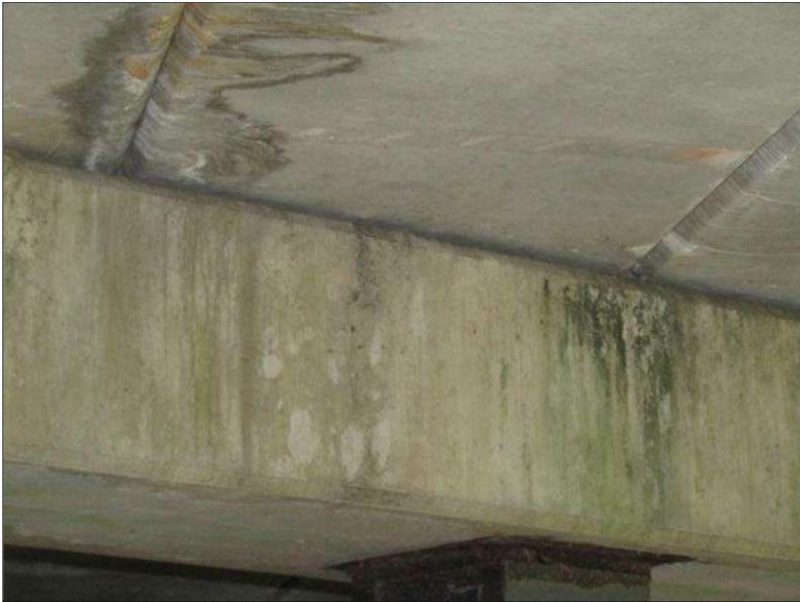
Span 3 Expansion Joint: OLD MOISTURE SEEPAGE STAIN ON PIER 2 CAP
