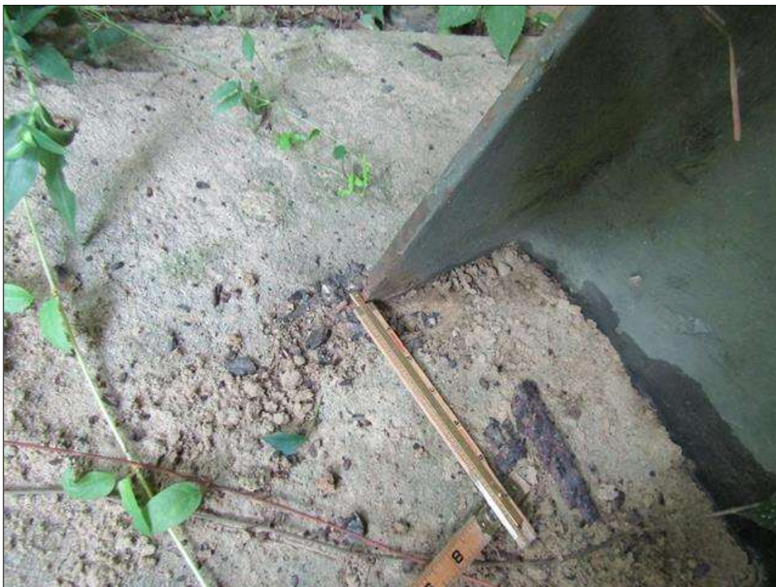
Bent 1 Pile 6: RUST SCALE ON PILE PLATE WITH SURFACE RUST ON TOP AND RUST SCALE ON BOTTOM OF FLANGE ON BOTH EAST SIDES WITH 7/16" STEEL REMAINING ON 1/2" FLANGE
