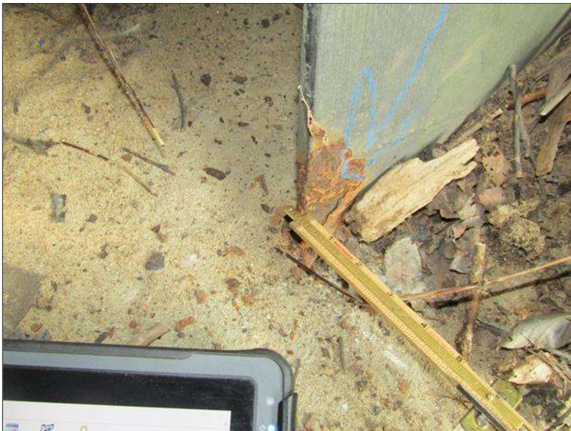
Bent 2 Pile 6: RUST SCALE ON BOTTOM OF SOUTH FLANGE ON WEST SIDE UP 3" X 2" WIDE WITH 1/4" STEEL REMAINING ON 1/2" FLANGE/PAR
