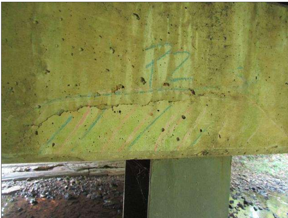
Bent 2 Cap 1: DELAM AREA ON NORTH FACE OVER PILE 2, 18" LONG X 5" WIDE
