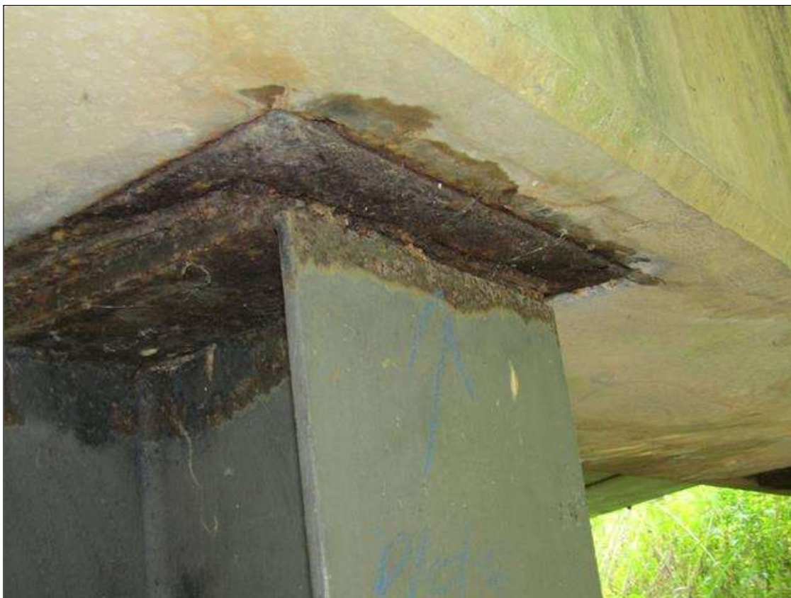
Bent 2 Pile 5: RUST SCALE ON TOP PLATE WITH SURFACE RUST ON TOP OF PILE
