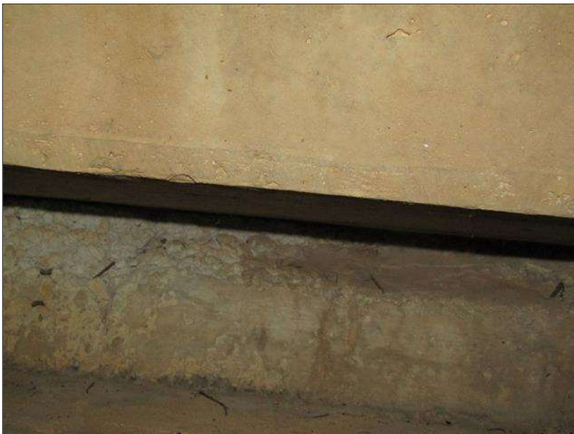
End Bent 1 Abutment: CONCRETE VOIDS IN TOP WHERE CONCRETE WAS POURED BETWEEN PILES 1-4
