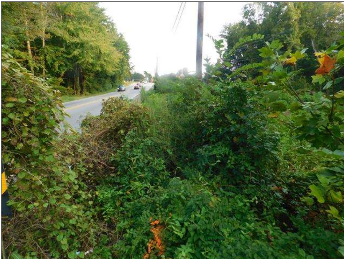
THICK BRUSH GROWING ON EAST SIDE OF BRIDGE
