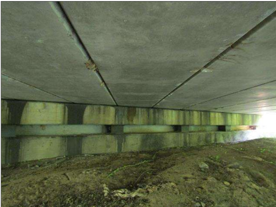
Span 3 Expansion Joint: OLD MOISTURE STAIN ON END BENT 2 CAP
