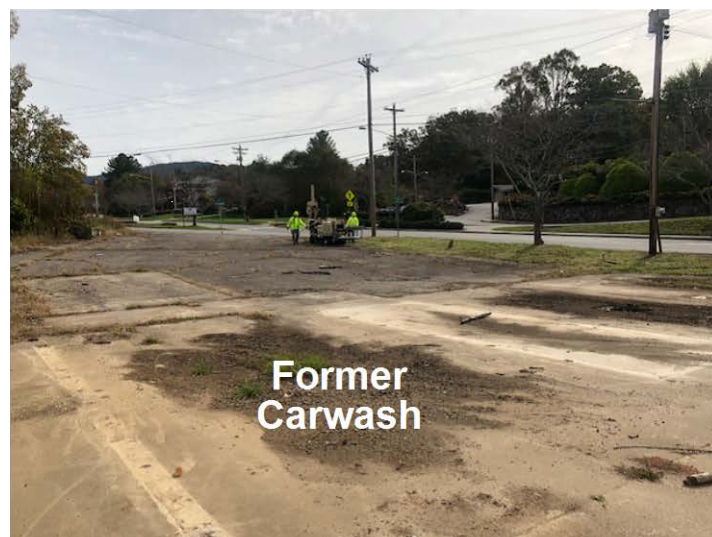
Drillers setting up on boring B-17. Footprint of former carwash is in the foreground.
