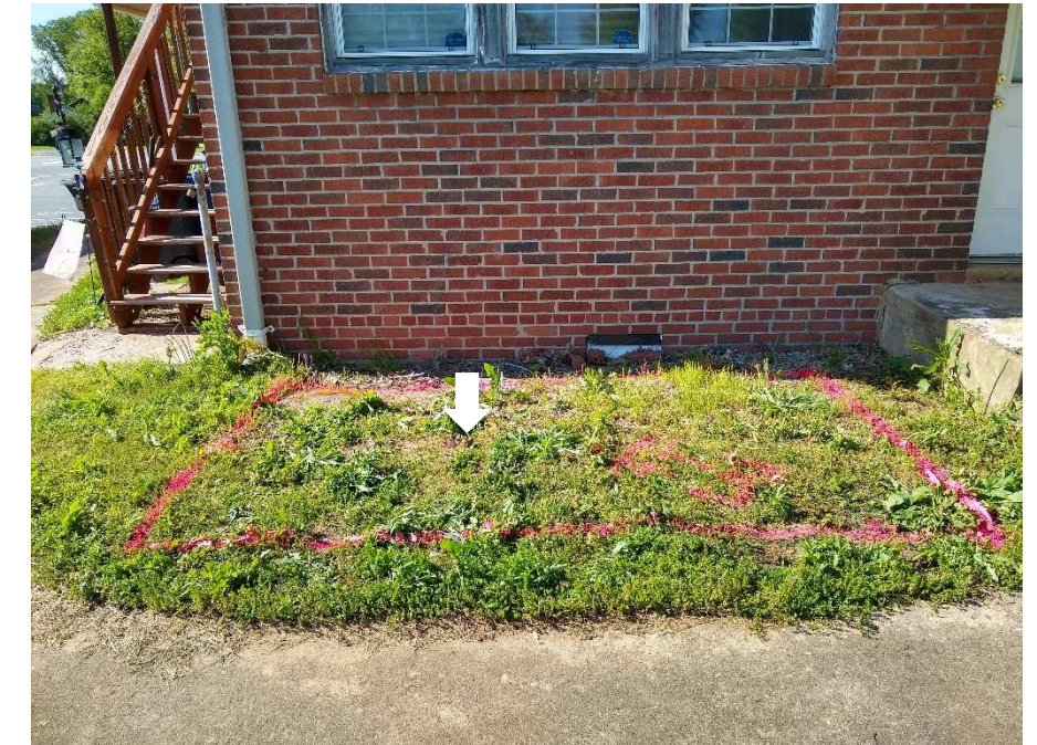
F. Photograph of rear of residence showing marked location of probable abandoned heating oil UST with apparent vent or fill pipe indicated by white arrow.
