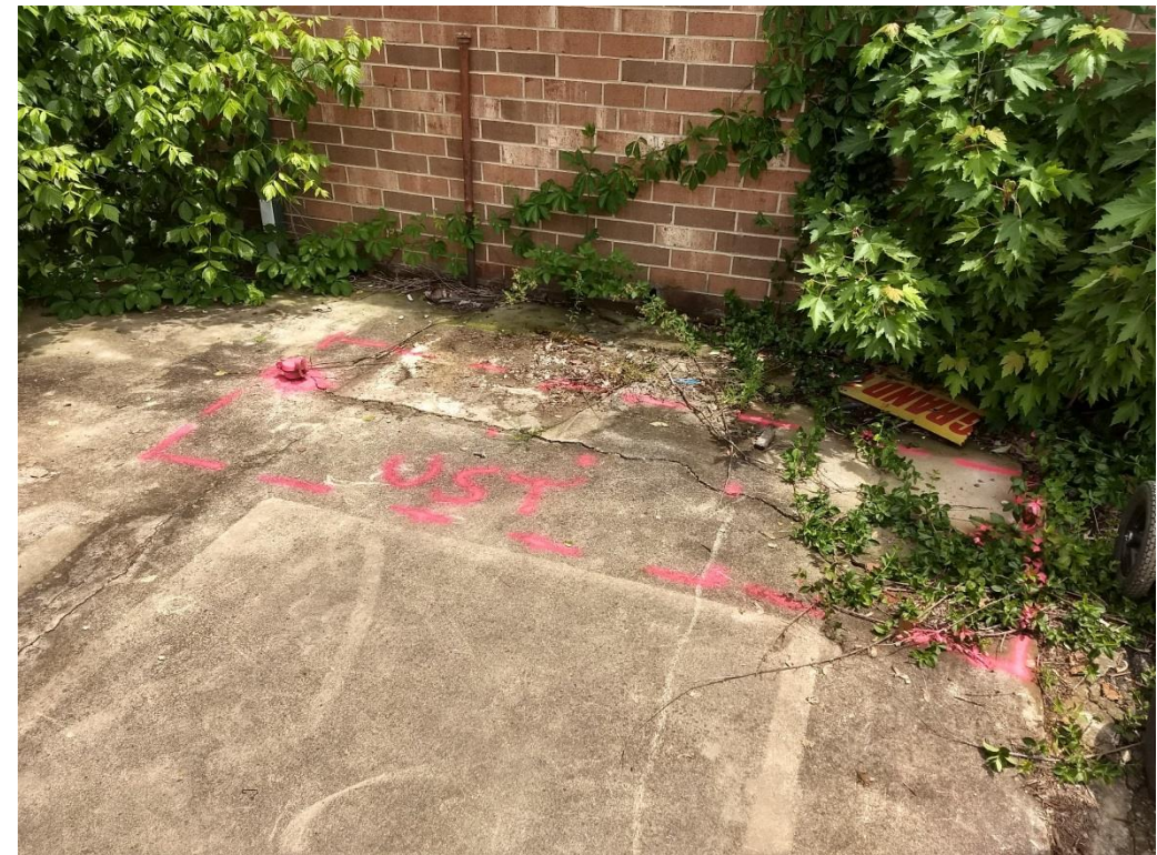
d. Photo of marked probable UST.
