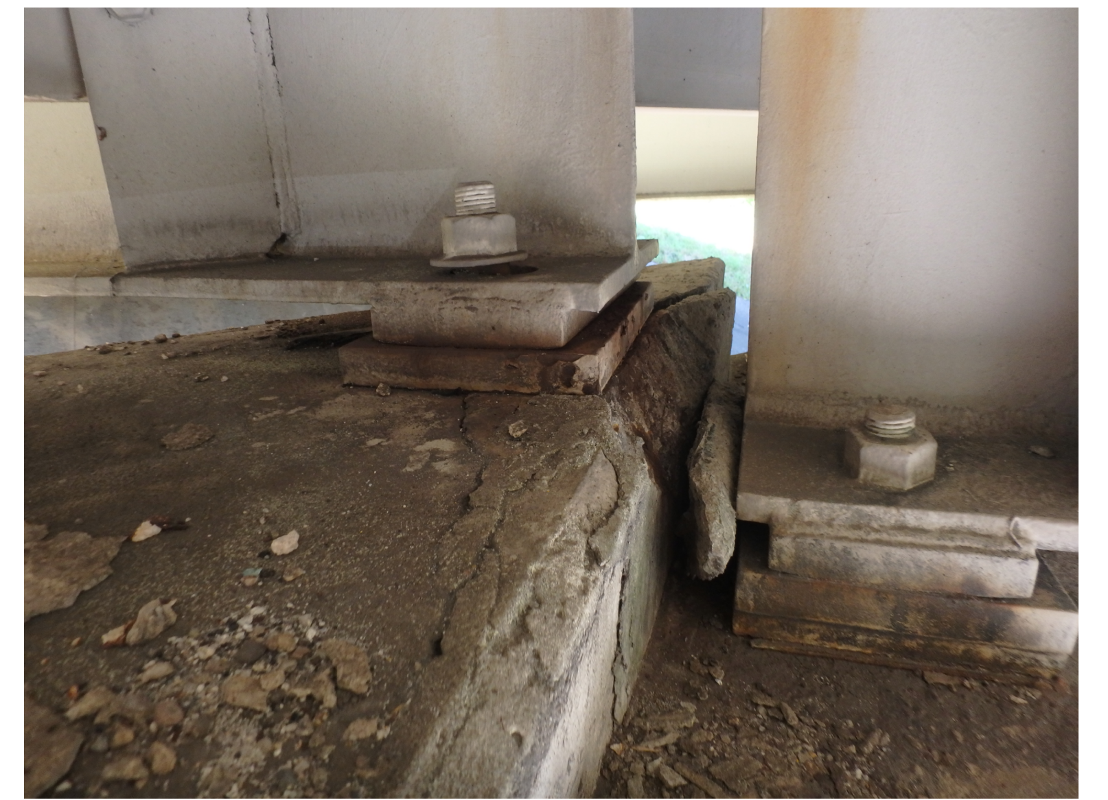
TYPICAL PEDESTAL CONDITION
