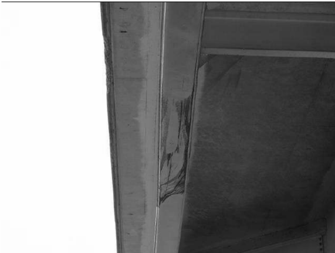
Span 2 Beam 1: IMPACT DAMAGE WITH 1/2" OF DISTORTION IN WEB AND BOTTOM FLANGE
