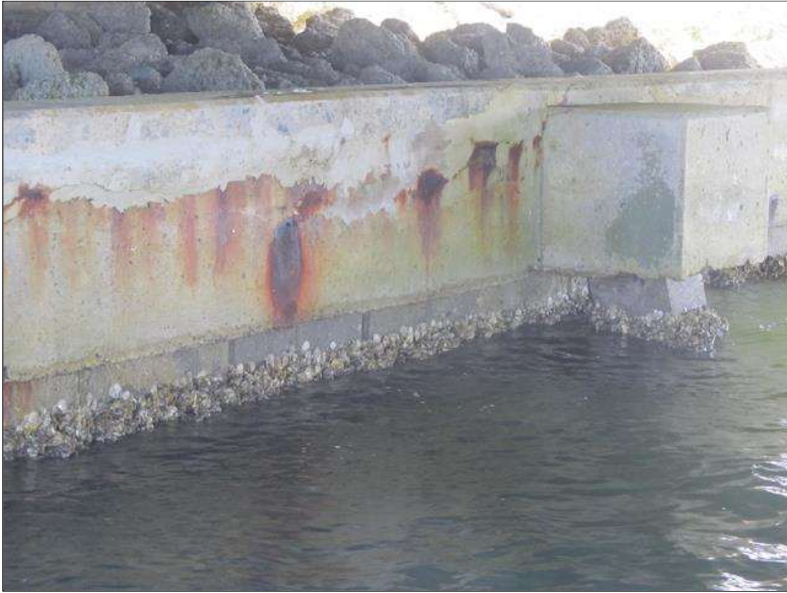
SIMILAR SEAWALL IN SPAN 12 WITH UNSOUND PATCHING, CRACKING & RUST STAINING.
