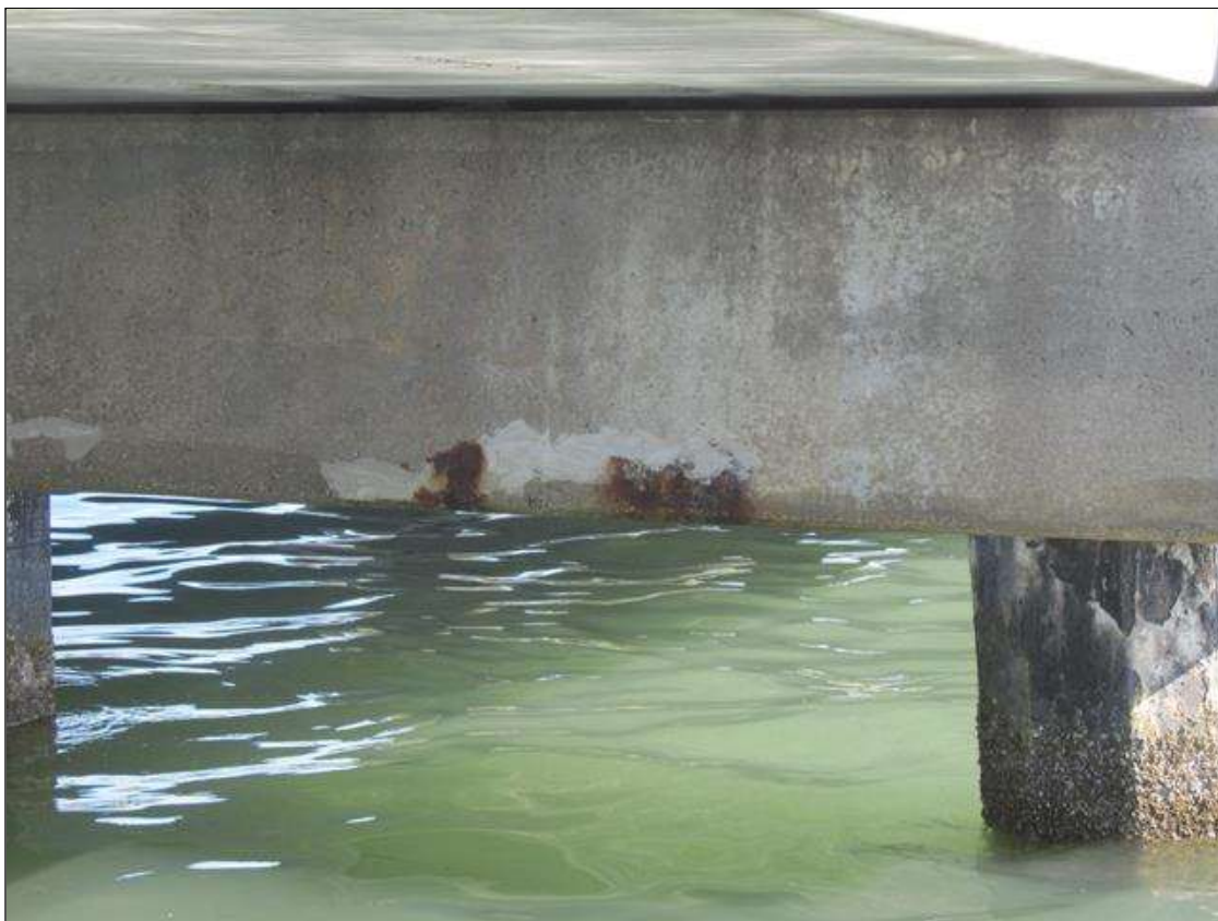
Bent 7 Cap 1: 33' OF POOR UNSOUND PATCHING WITH CRACKING & RUST STAINING ALONG THE CAP.
