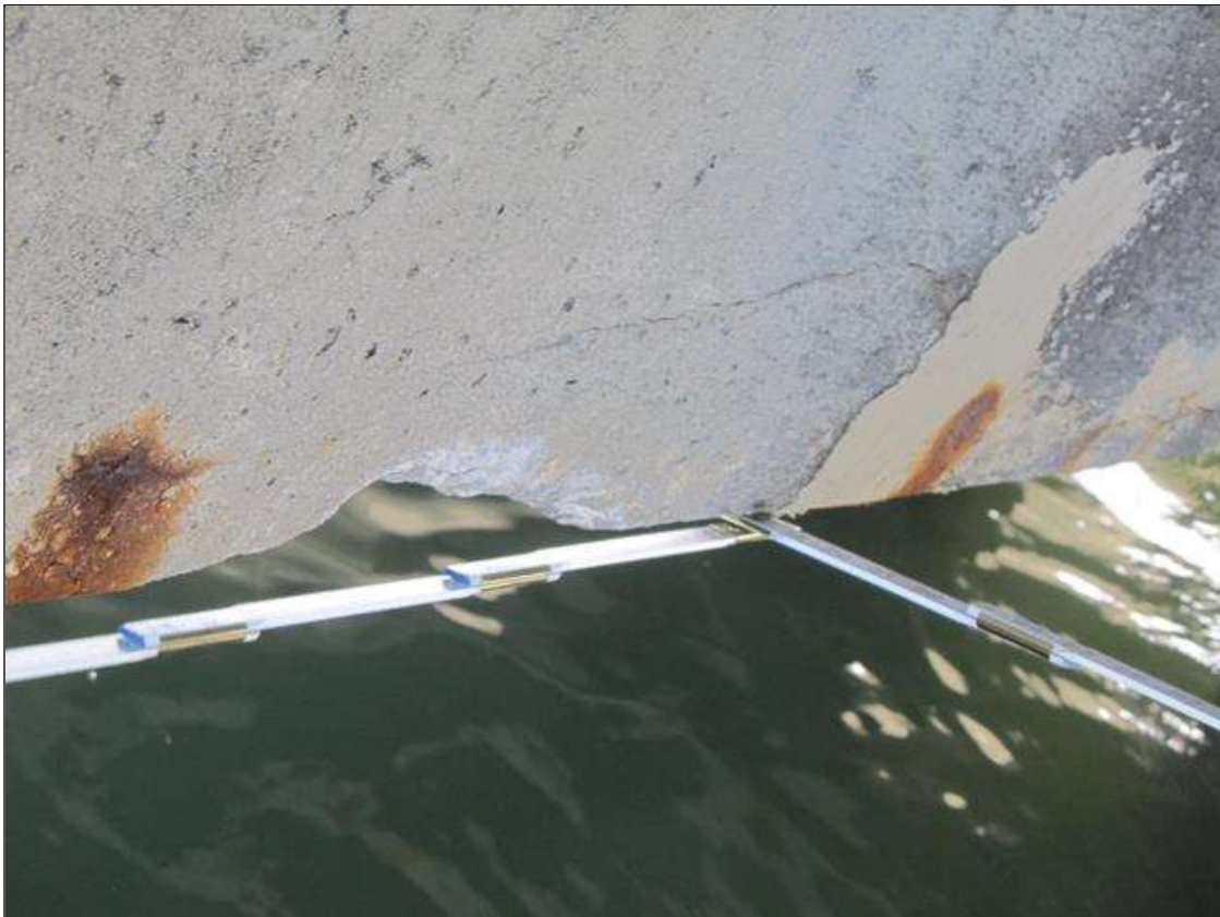
Bent 4 Cap 1: 2' OF POOR SPALL TO 8" L X 3" H X 4" W AND DELAMINATION TO 13" L X 3" H X 4" W @ THE BOTTOM EDGE NEAR PILE 1
