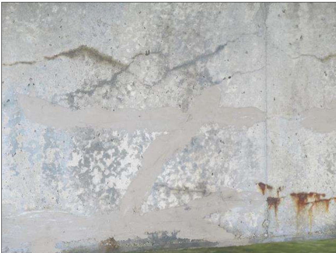
Bent 10 Cap 1: 31' OF POOR CRACKING & UNSOUND PATCHES ALONG FACES.
