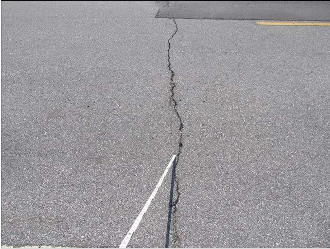
Span 1 Wearing Surface: 26 SQUARE FEET OF POOR TRANSVERSE CRACKING OVER END BENT 1.
