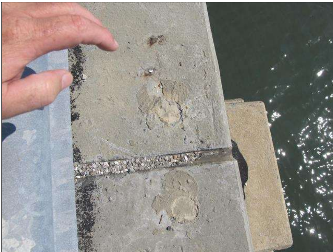
Expansion Joint : 4 FEET OF FAIR DEBRIS AT THE EXPOSED PORTIONS IN THE RIGHT & LEFT SHOULDERS.
