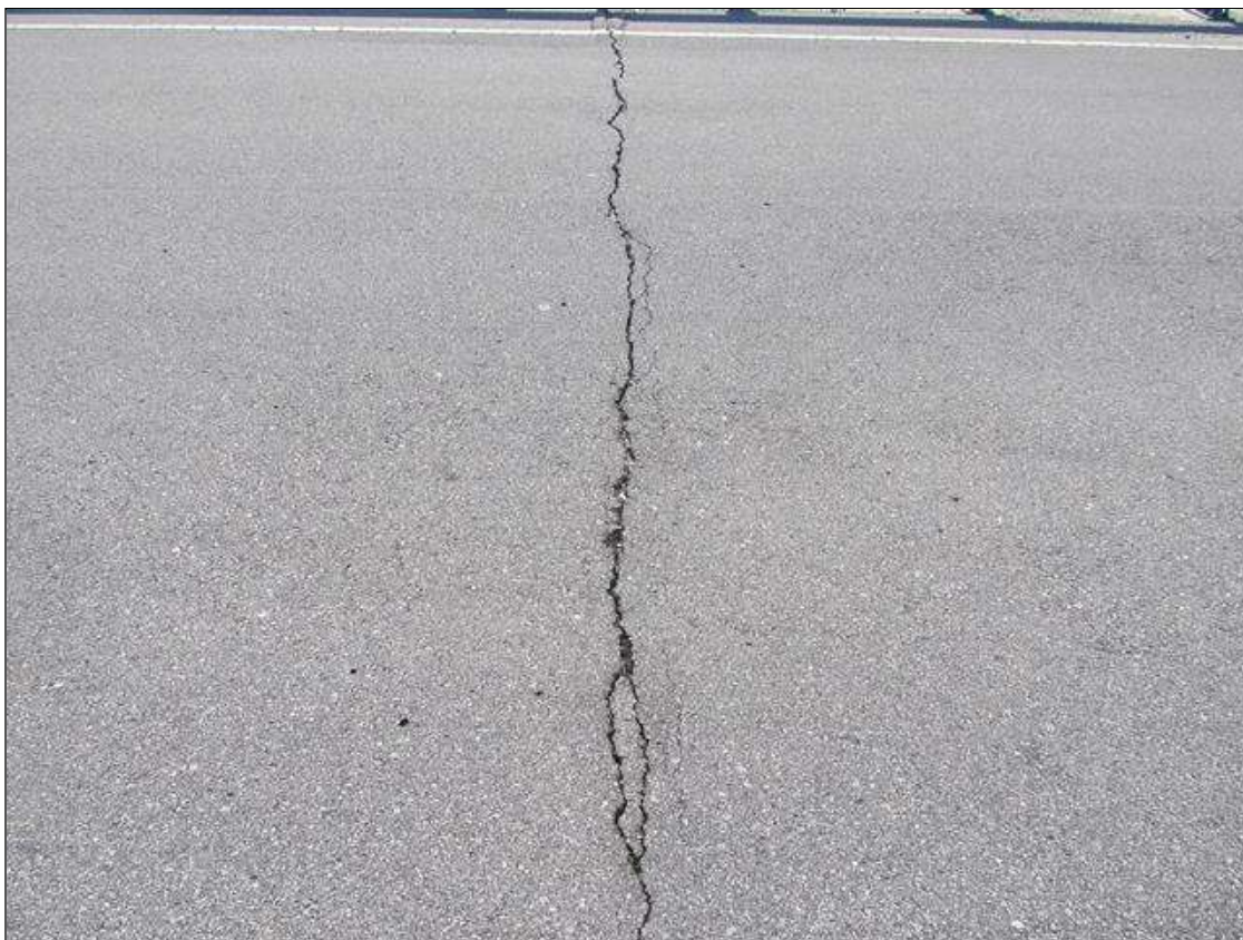
Span 2 Wearing Surface: 26 SQUARE FEET OF POOR TRANSVERSE CRACKING OVER BENT 1. SIMILAR OVER ALL INTERIOR BENTS.
