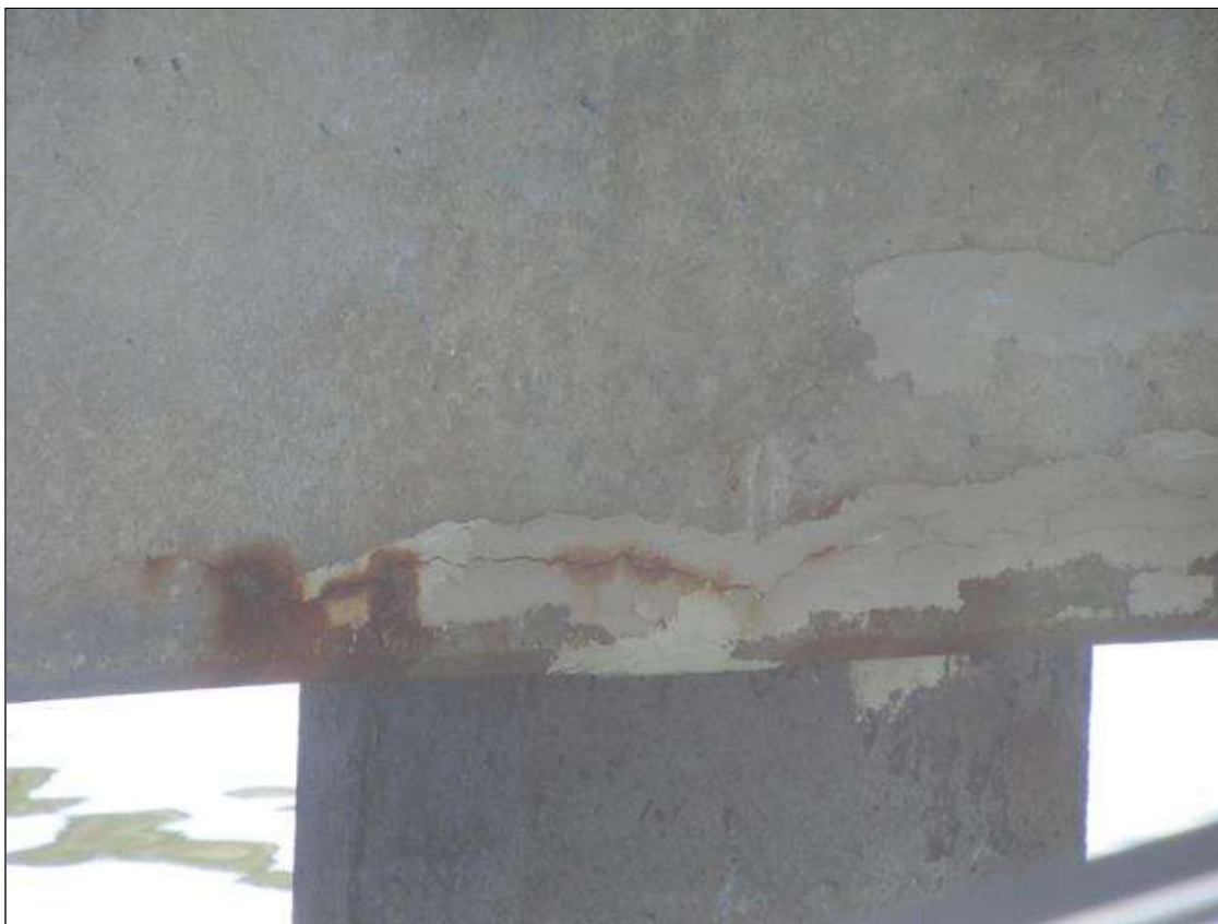
Bent 11 Cap 1: 33' OF POOR UNSOUND PATCHING WITH CRACKING & RUST STAINING ALONG THE CAP.
