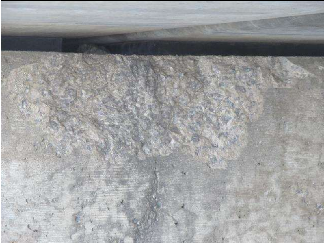
Bent 1 Cap 1: 2' OF POOR SPALL TO 20" L X 6" H X 1" DEEP IN SPAN 1 FACE @ THE TOP CORNER BETWEEN SLABS 1 & 2
