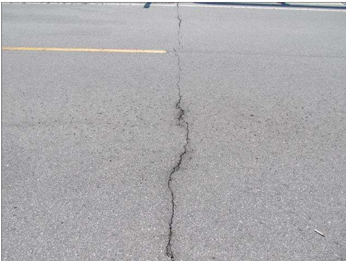
Span 13 Wearing Surface: 26 SQUARE FEET OF POOR TRANSVERSE CRACKING OVER END BENT 2.
