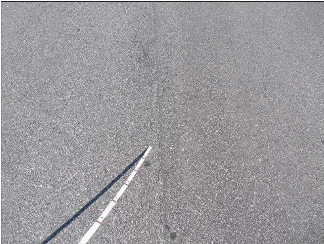
Span 2 Wearing Surface: 25 SQUARE FEET OF FAIR LONGITUDINAL CRACKING IN SHOULDERS & LANES.
