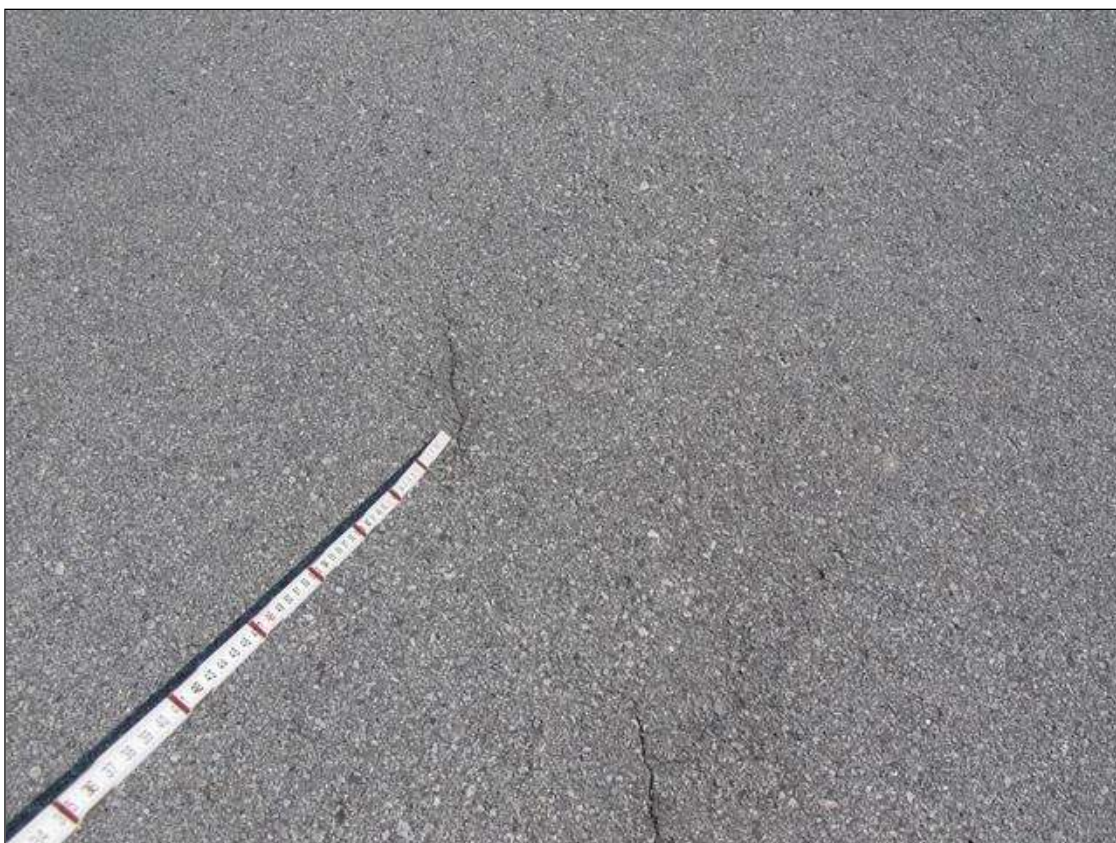
Span 6 Wearing Surface: 20 SQUARE FEET OF POOR LONGITUDINAL IN LANES & SHOULDERS.
