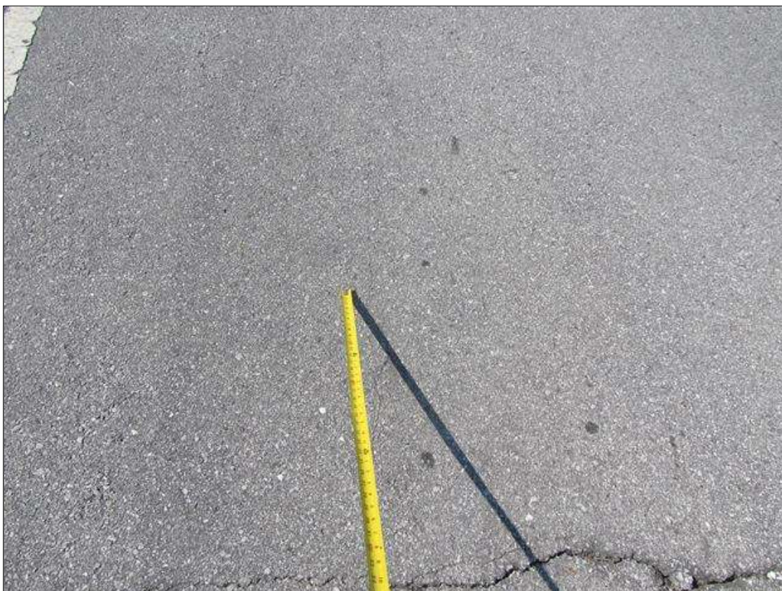
Span 3 Wearing Surface: 12 SQUARE FEET OF FAIR LONGITUDINAL CRACKING IN THE RIGHT SHOULDER NEAR BENTS.
