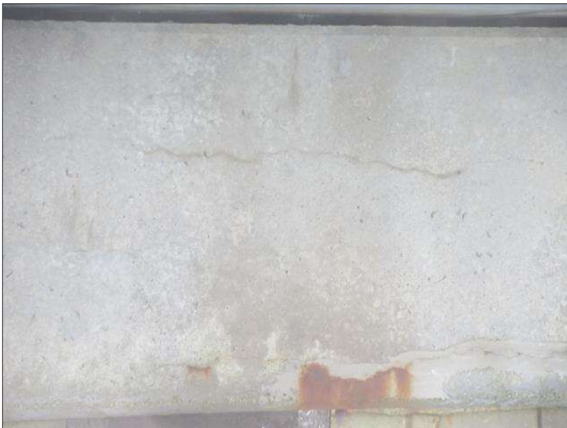
Bent 12 Cap 1: 33' OF POOR UNSOUND PATCHING WITH CRACKING & RUST STAINING ALONG THE CAP.
