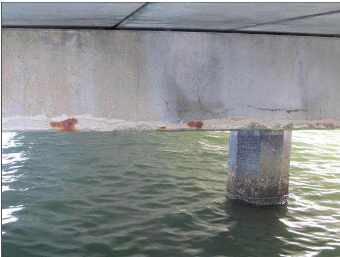
Bent 5 Cap 1: 33' OF POOR UNSOUND PATCHING WITH CRACKING & RUST STAINING ALONG THE CAP.
