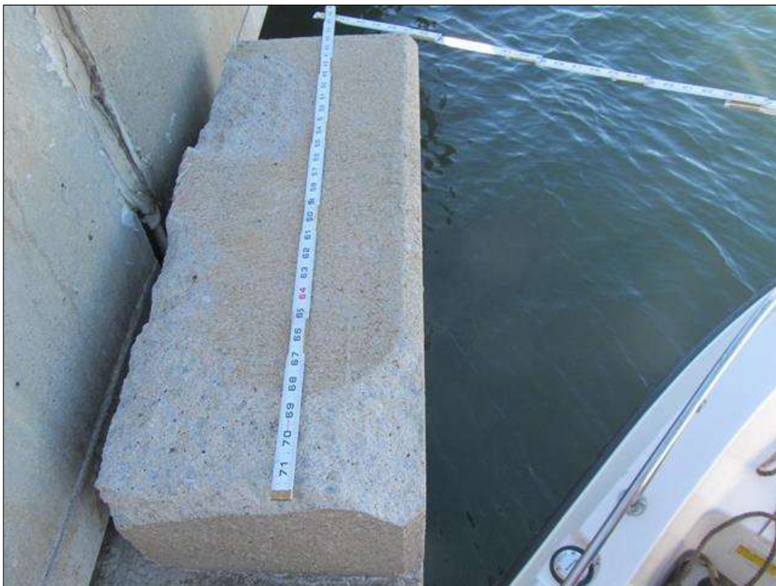
Bent 10 Cap 1: 2' OF POOR SPALL IN THE TOP LEFT RETAINING BLOCK TO 28" LONG X 6- 10" WIDE X 1/2- 3/4" DEEP
