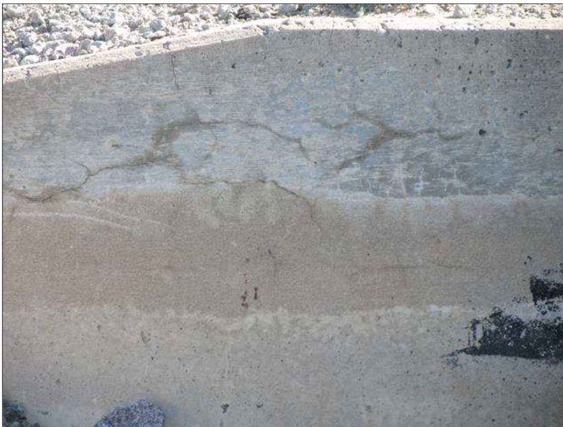
End Bent 2 Abutment/Backwall : 4' OF FAIR CRACKING @ THE LEFT EXTERIOR.
