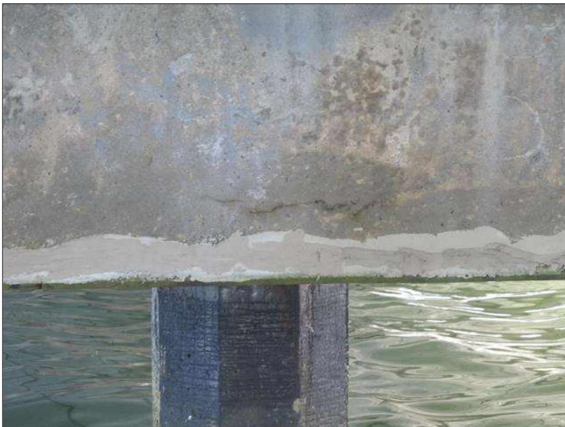
Bent 6 Cap 1: 33' OF POOR UNSOUND PATCHING WITH CRACKING BLEEDING THRU & UNSEALED.
