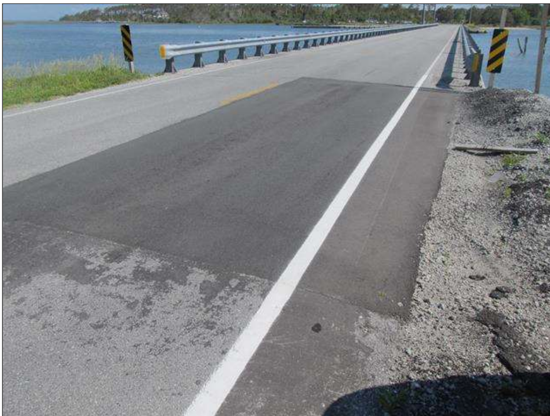
SOUTH APPROACH ROADWAY PATCHED IN THE RIGHT LANE & SHOULDER TO 30' LONG X 12' PAVED & 6' SHOULDER WIDE.
