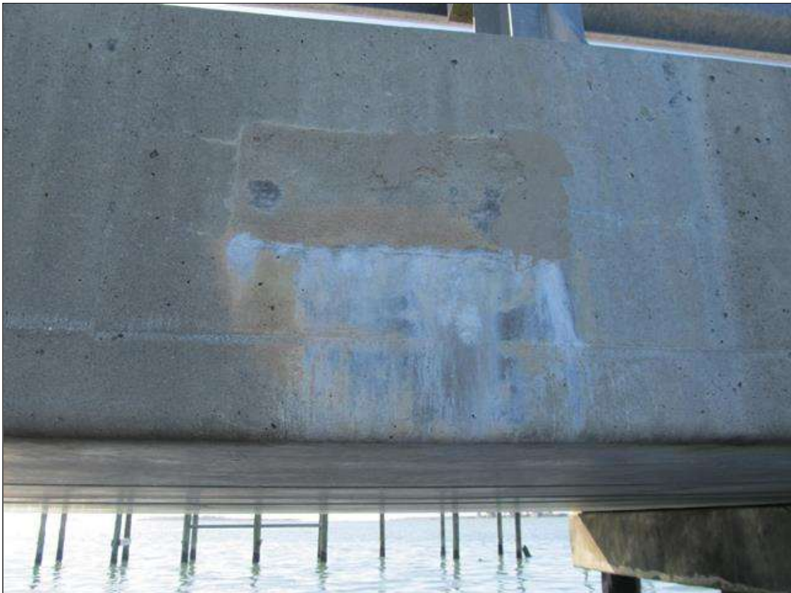
Span 2 Slab 1: 1 FOOT OF POOR EFFLORESCENCE @ THE 1/3 TRANSVERSE CABLE PORT.
