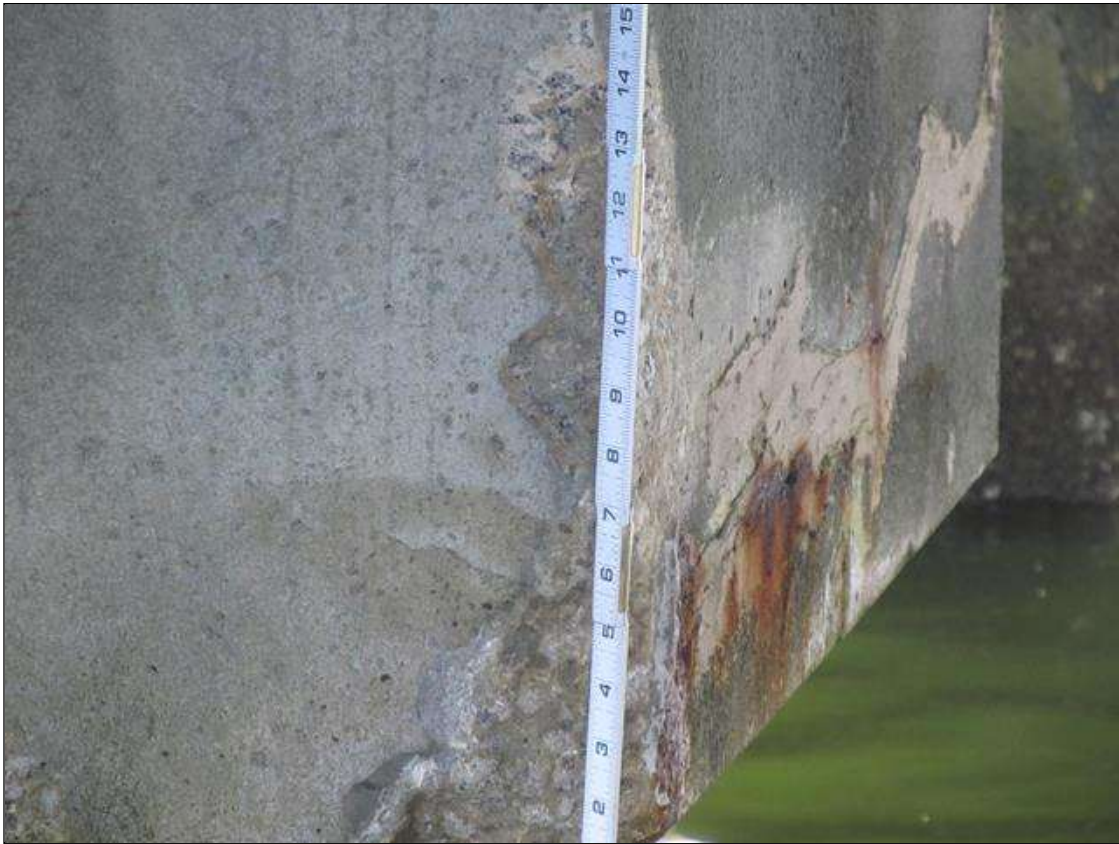
Bent 4 Cap 1: 6' OF POOR CROSS CAPS @ BENT 4 WITH UNSOUND PATCHES, RUST STAINS & SPALL ON SOUTHWEST CORNER OF CROSSCAP 1 TO 14" HIGH X 4" WIDE.
