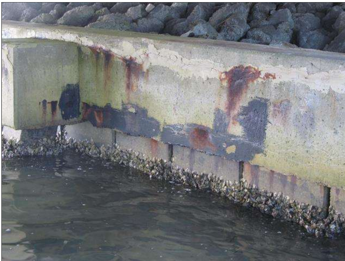
SIMILAR SEAWALL IN SPAN 1 WITH UNSOUND PATCHING, CRACKING & RUST STAINING.
