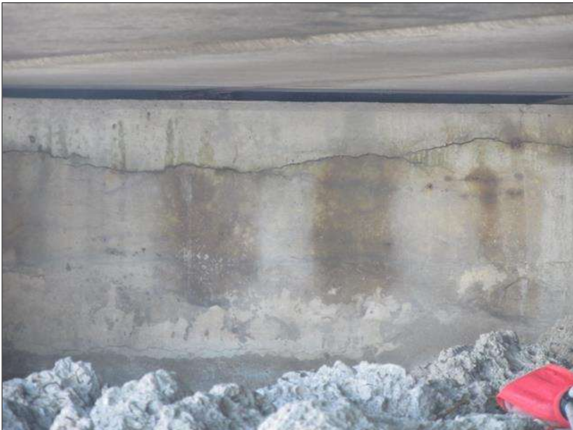
End Bent 2 Cap 1: 33' OF POOR CRACKING ALONG THE SOUTH FACE.
