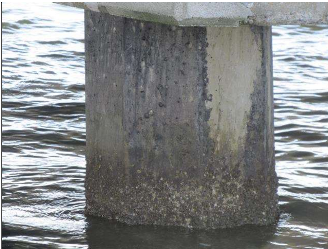
Bent 4 Pile 1: 6' OF FAIR SEALED CRACKS @ THE SOUTH FACE, SOUTHWEST FACE & WEST FACE.
