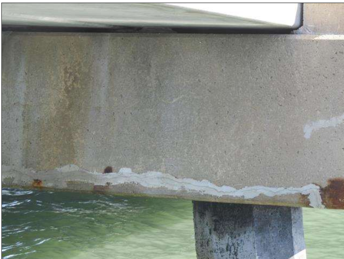
Bent 8 Cap 1: 33' OF POOR UNSOUND PATCHING WITH CRACKING & RUST STAINING ALONG THE CAP.
