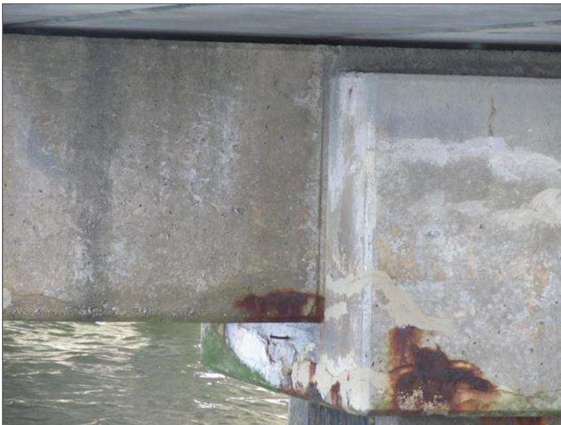
Bent 9 Cap 1: 33' OF POOR UNSOUND PATCHING WITH CRACKING & RUST STAINING ALONG THE CAP.
