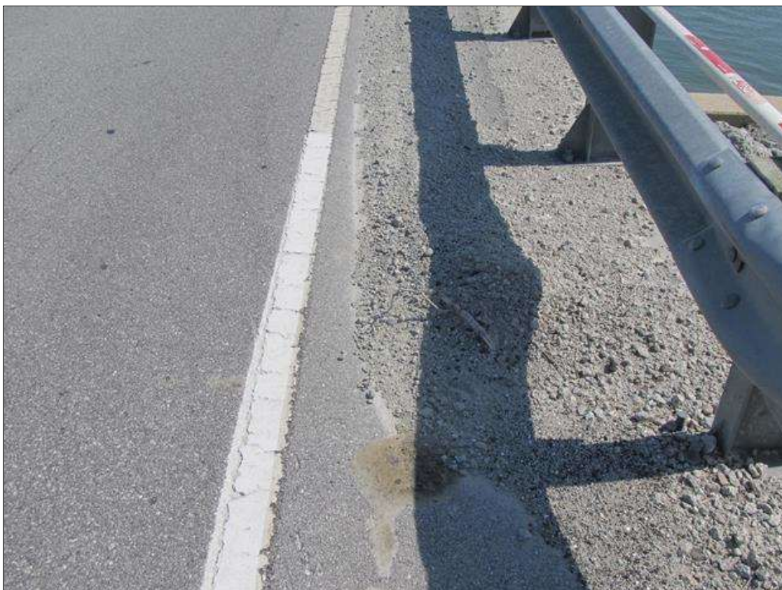
DEBRIS AT SHOULDERS.
