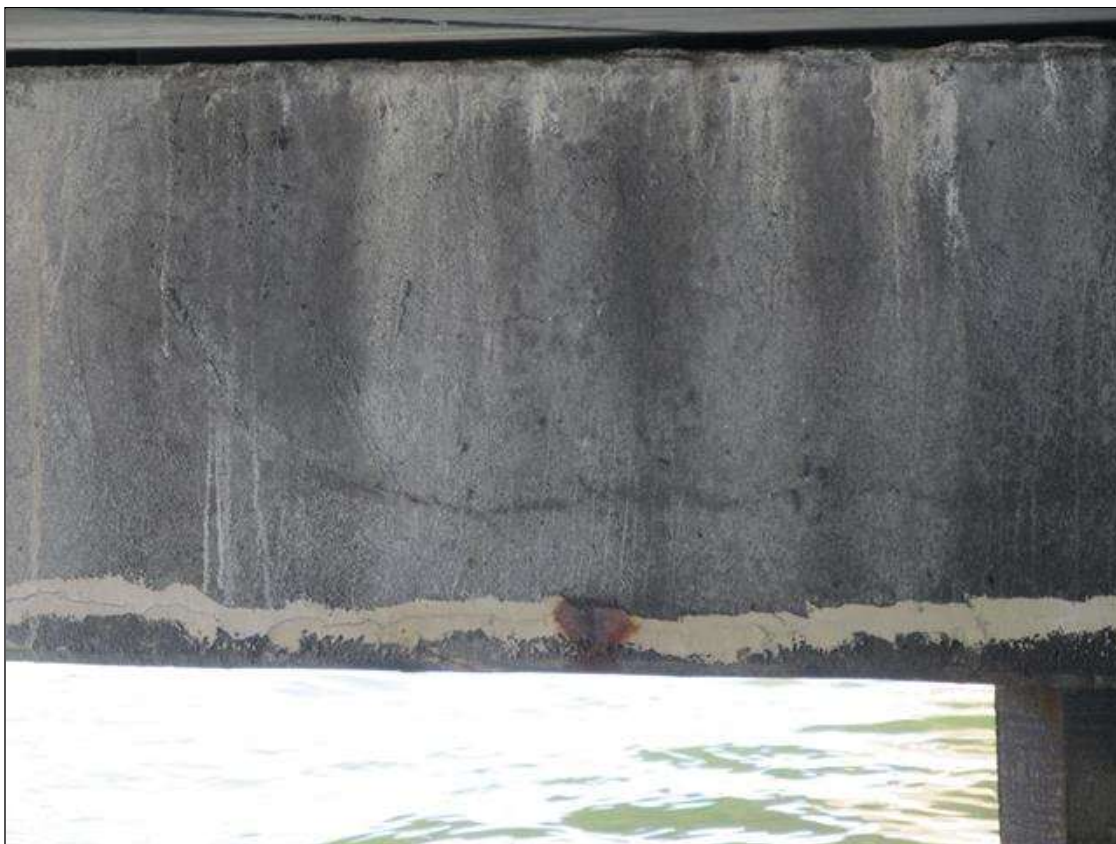
Bent 2 Cap 1: 33' OF POOR UNSOUND PATCHING WITH CRACKING & RUST STAINING ALONG THE CAP.
