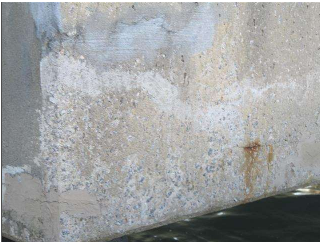
Bent 3 Cap 1: 33' OF POOR UNSOUND PATCHING WITH CRACKING & RUST STAINING ALONG THE CAP.
