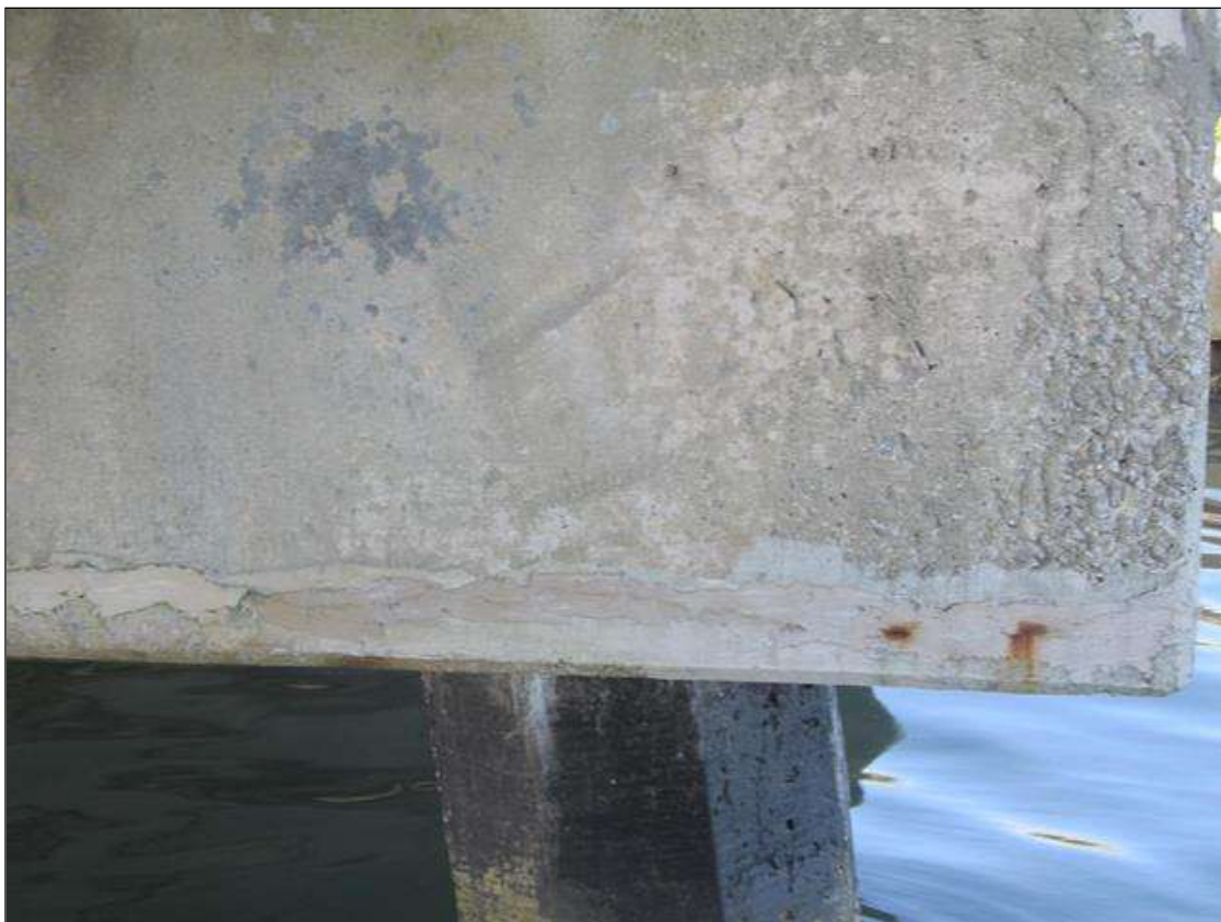
Bent 1 Cap 1: 31' OF POOR UNSOUND PATCHING WITH CRACKS & ALONG THE LOWER PORTIONS & ENDS OF
