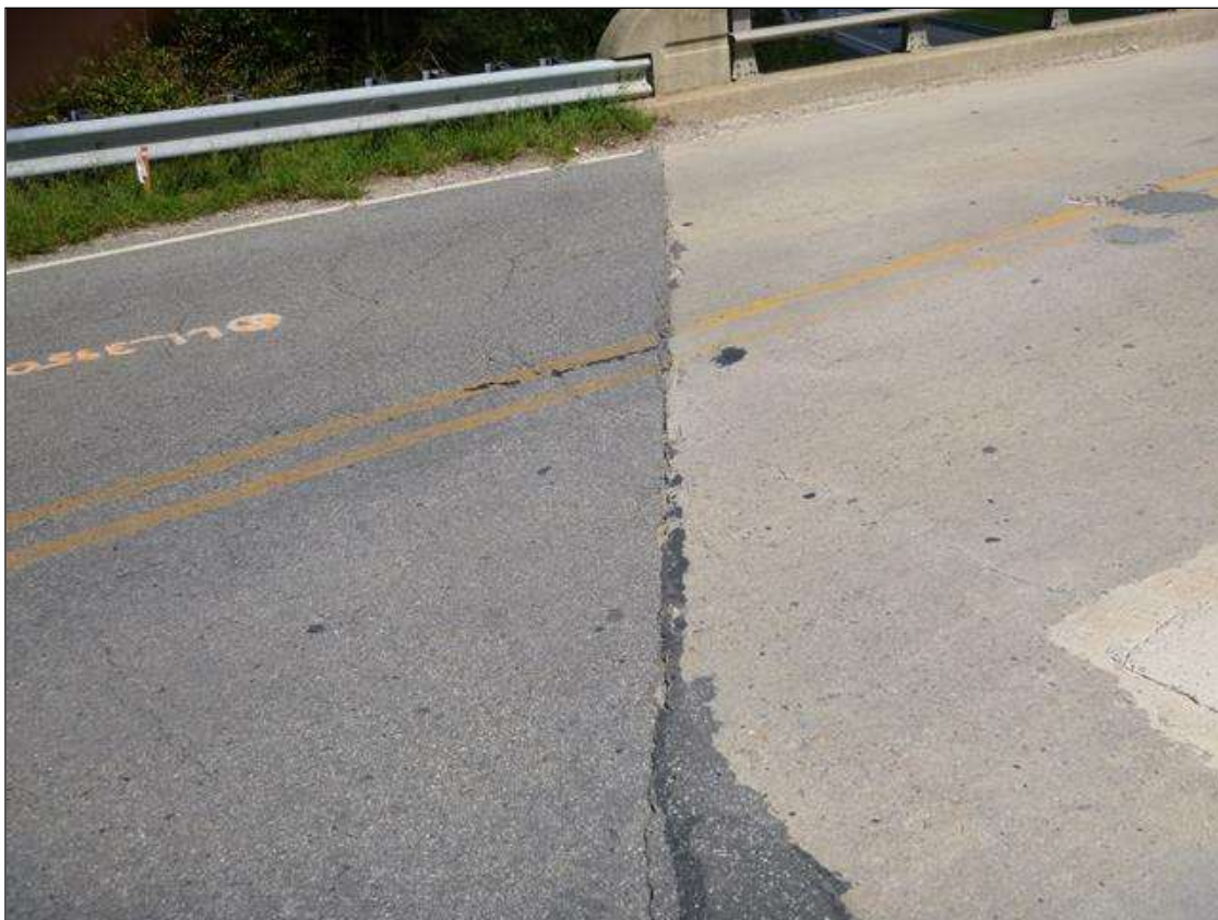
CRACK OVER END BENT 1, LOOKING NORTH
