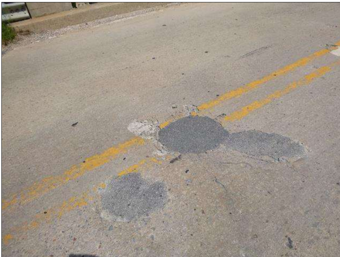
Span 1 Deck: (2) 1 FT DIAMETER ASPHALTIC PATCHES, AT CENTERLINE, 10 FEET FROM END BENT 1.
