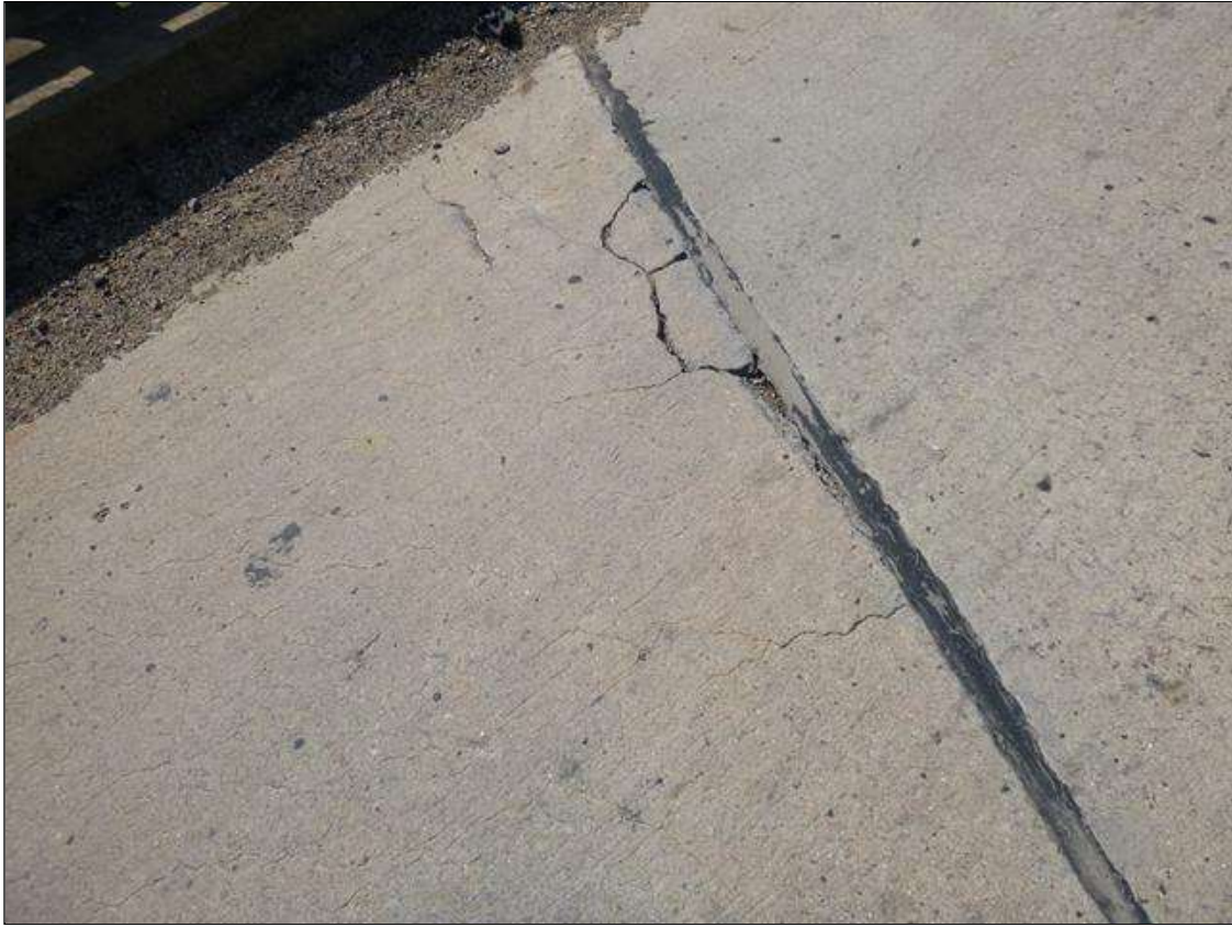
Expansion Joint, Bent 3 : 18" X 5" DELAMINATION, ALONG SPAN 4 HEADER, NEAR SOUTH CURB.
