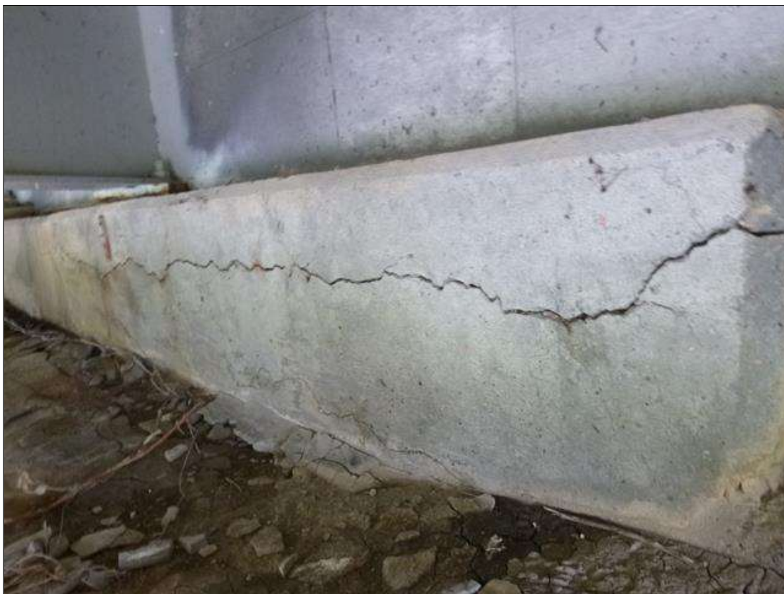
End Bent 5 Cap 1: 5 FT HORIZONTAL CRACK UP TO 1/8 IN, BELOW BAY 3.
