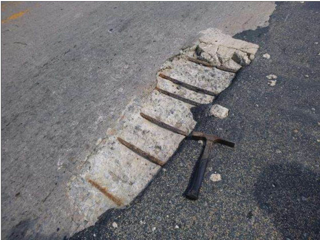
Span 1 Deck: 4' X 18" X 2" DEEP SPALL WITH EXPOSED REINFORCING, CENTER OF EAST BOUND LANE, NEAR MIDSPAN. (PM)
