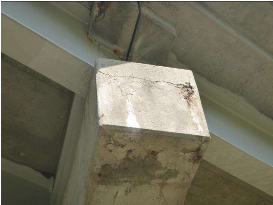
Bent 4 Cap 1: 3 FT X 3 FT AREA OF SPALLING AND DELAMINATION, SOUTH FACE OF BENT CAP.
