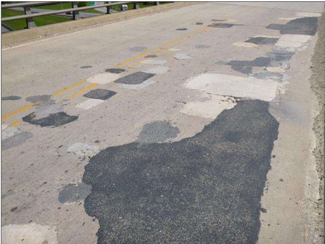
Span 2 Deck: 350 SQ FT AREA OF SOUND AND UNSOUND PATCHES THROUGHOUT EASTBOUND LANE.
