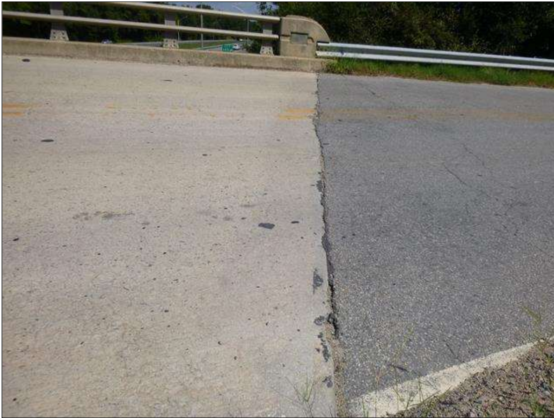
CRACK OVER END BENT 2, LOOKING NORTH
