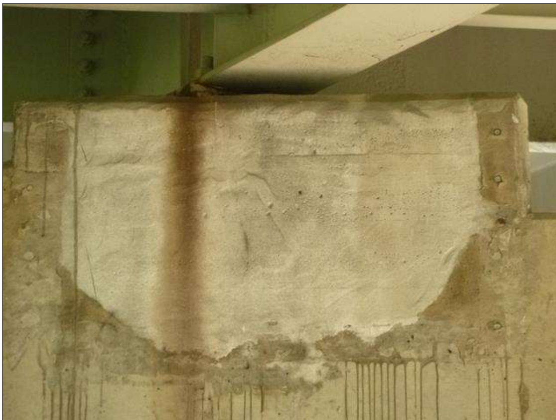
Bent 1 Cap 1: 30" X 2' SOUND PATCHED AREA, WEST FACE BELOW BEAM 3.
