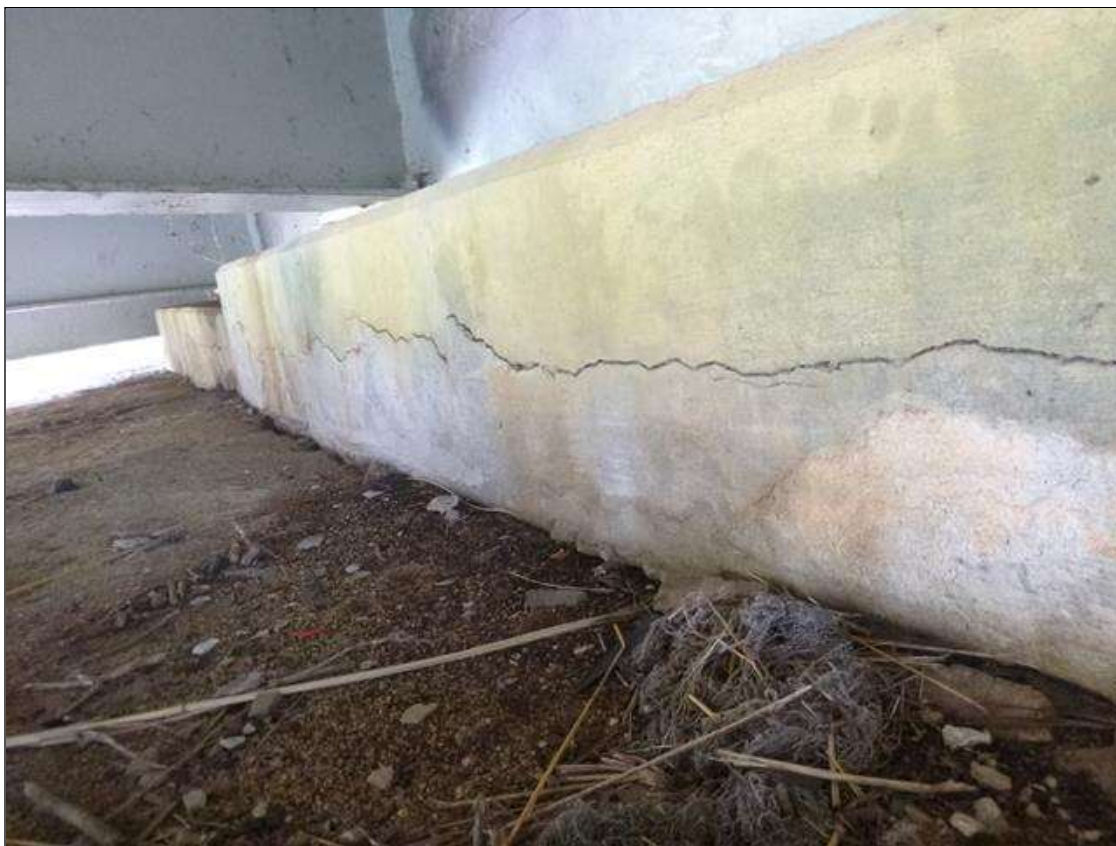
End Bent 1 Cap 1: 20 FT HORIZONTAL CRACK UP TO 1/8 IN, BETWEEN BEAMS 1 THROUGH 4.
