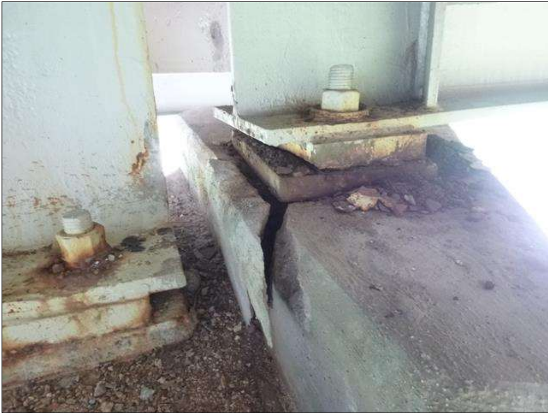
Bent 1 Cap 1: 15" X 7'X 3" SPALL, EAST FACE OF SPAN 1 BEAM 2 SEAT. NO LOSS OF BEARING AREA.
