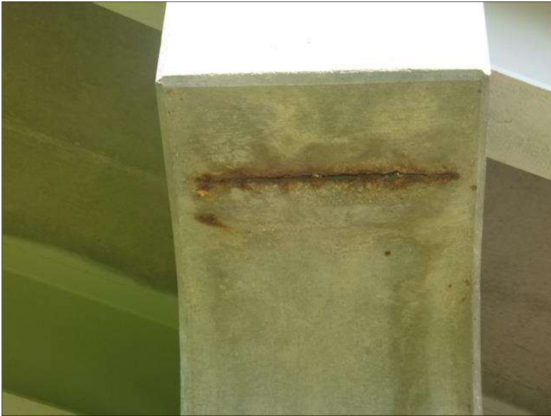
Bent 3 Cap 1: 2 FT X 6 IN SPALL WITH EXPOSED REINFORCEMENT ON UNDERSIDE OF RIGHT END OF CAP.
