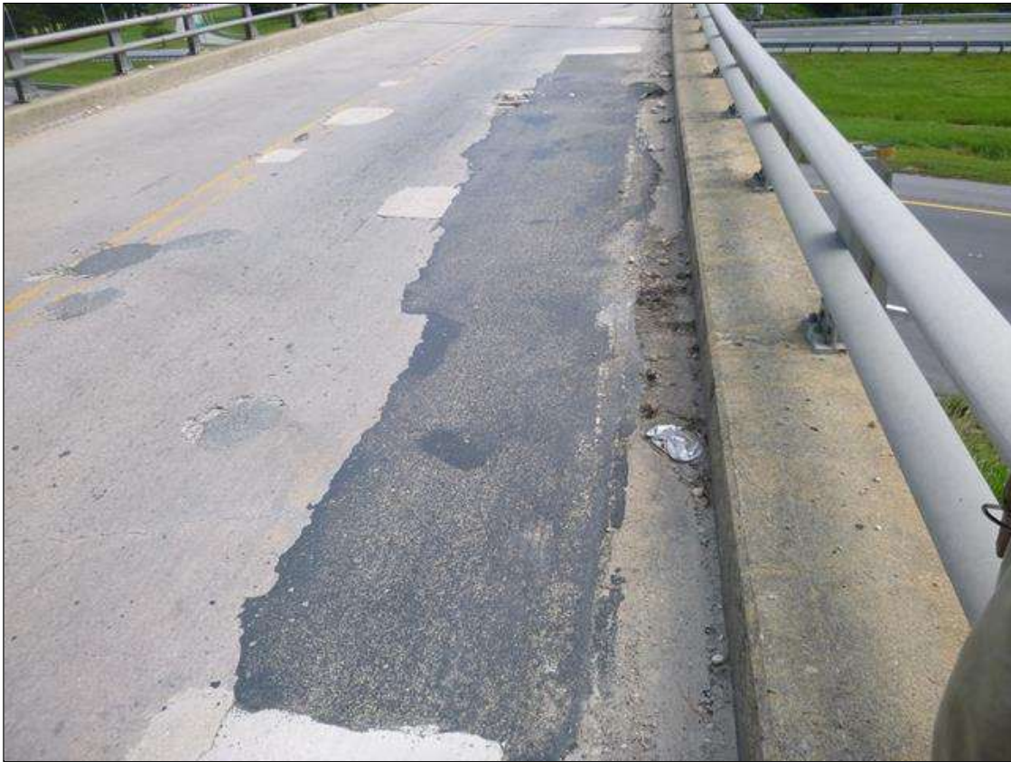
Span 1 Deck: 40 FT X 3 FT SOUND ASPHALTIC PATCH ALONG SOUTHERN PORTION OF EASTBOUND TRAVEL LANE.
