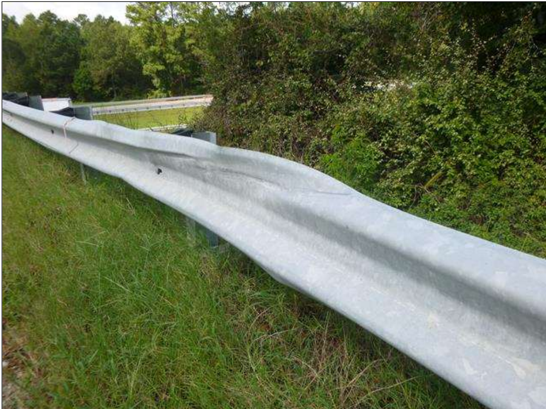
General Comments and Misc. Items: 8' OF IMPACT DAMAGE TO NORTHEAST GUARDRAIL.
