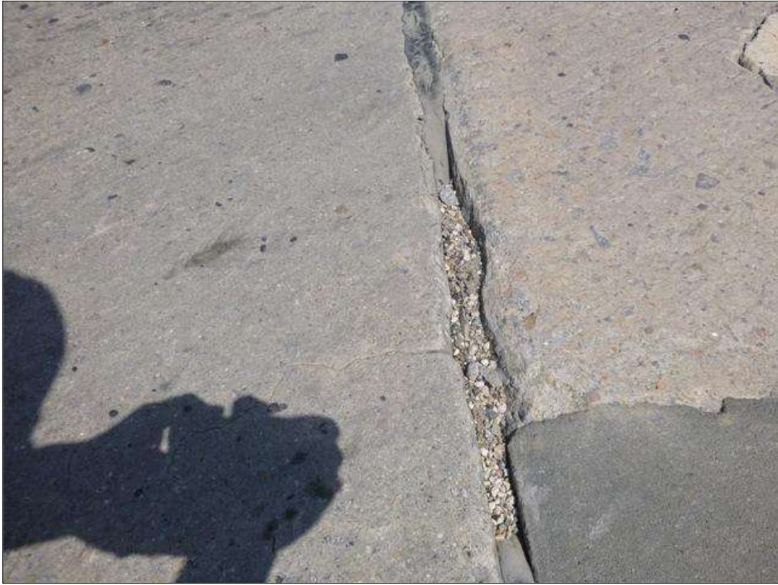
Expansion Joint, Bent 1 : 6' OF COMPLETE LOSS OF ADHESION AT RANDOM ALONG JOINT.
