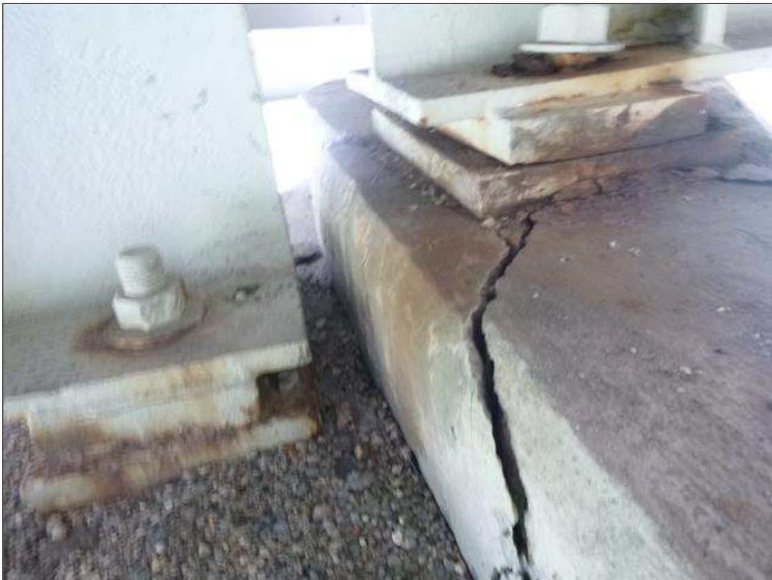
Bent 1 Cap 1: 20" X 6" DELAMINATION, EAST FACE OF SPAN 1 BEAM 3 SEAT.
