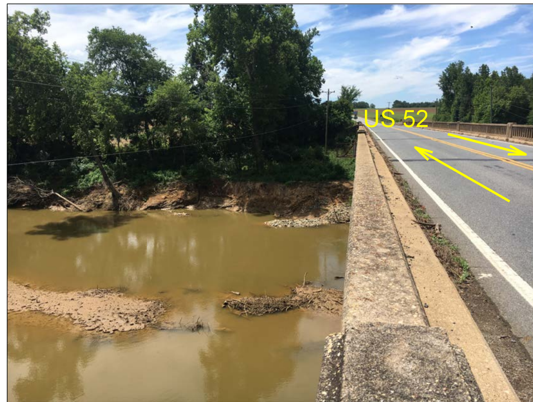
PHOTO 1: VIEW AT BENT 2 FACING DOWNSTATION ALONG PROPOSED NEW ALIGNMENT TOWARD END BENT 1.
