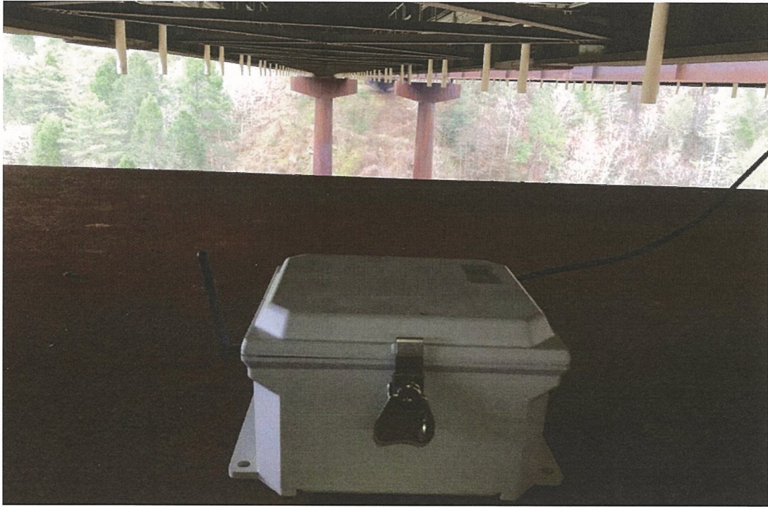
Figure 2. Sample Wireless Data Acquisition Gateway Attached to a Solar Panel (Not Shown)
