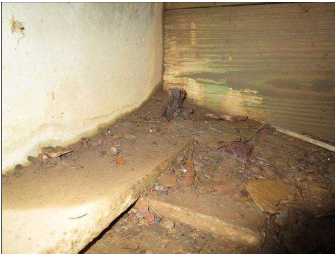
CORROSION TO VARIOUS ANCHOR BOLTS AT BOTH END BENTS
