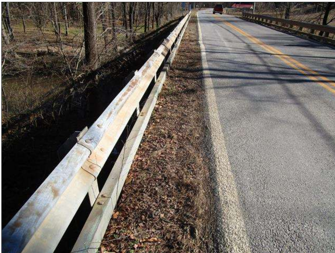
DEBRIS ALONG BOTH GUTTERLINES
