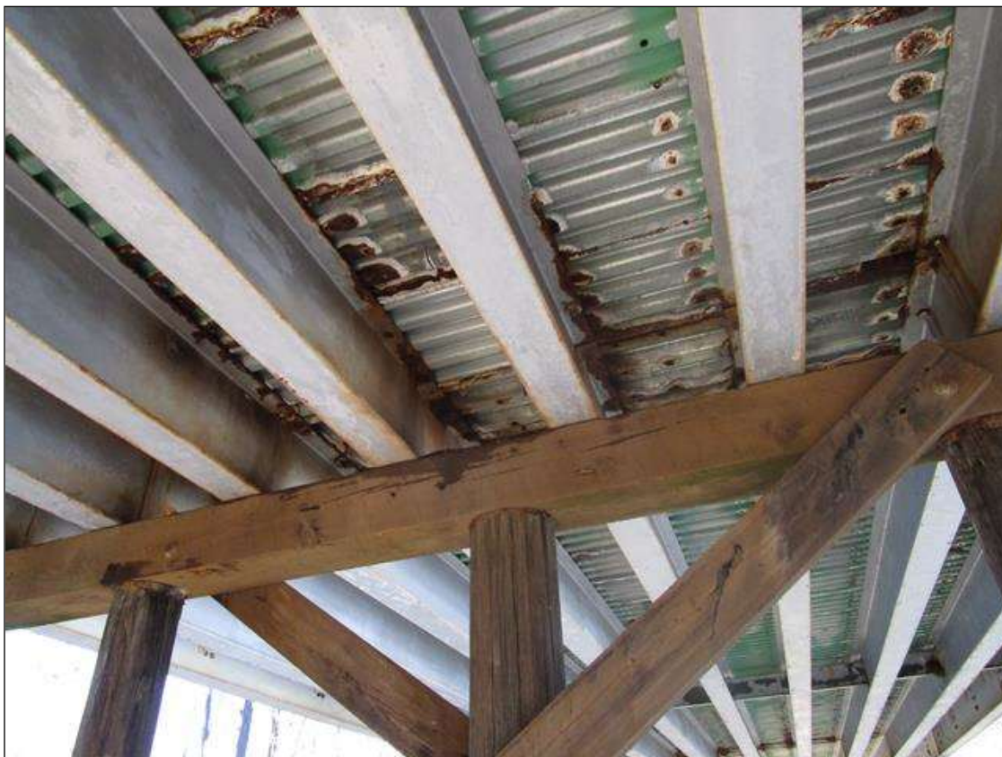
OVERVIEW OF CORROSION TO TOP FLANGES OF BEAMS 2-7 OVER BENT 1
