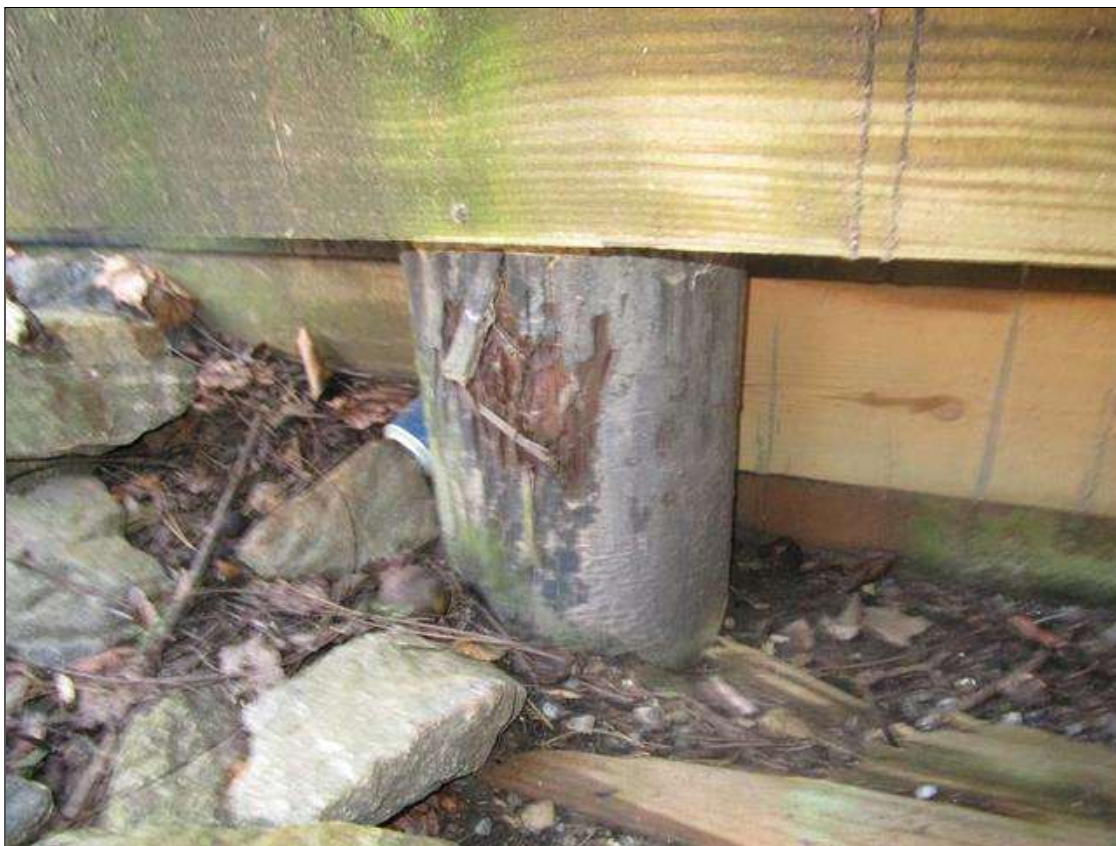
End Bent 2 Pile 1: 5" DIAMETER X 1" DEEP DECAY
