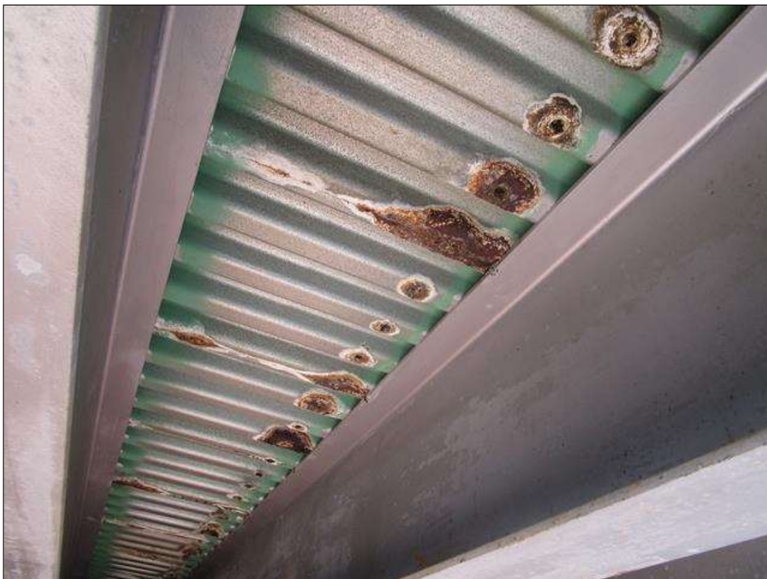
APPROXIMATELY 10% OF UNDERSIDE OF DECK IN ALL SPANS HAS CORROSION
