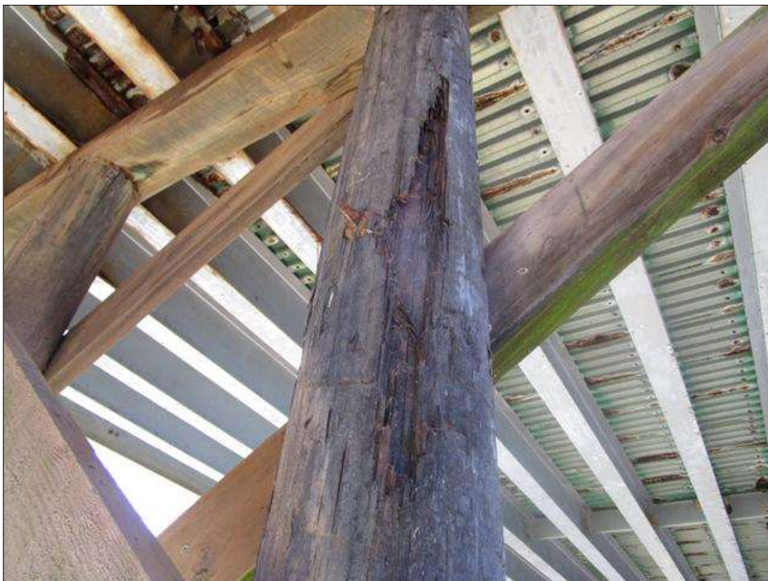
Bent 2 Pile 2: 2' HIGH X 3" WIDE X 0.5" DEEP DECAY IN NORTHEAST FACE
