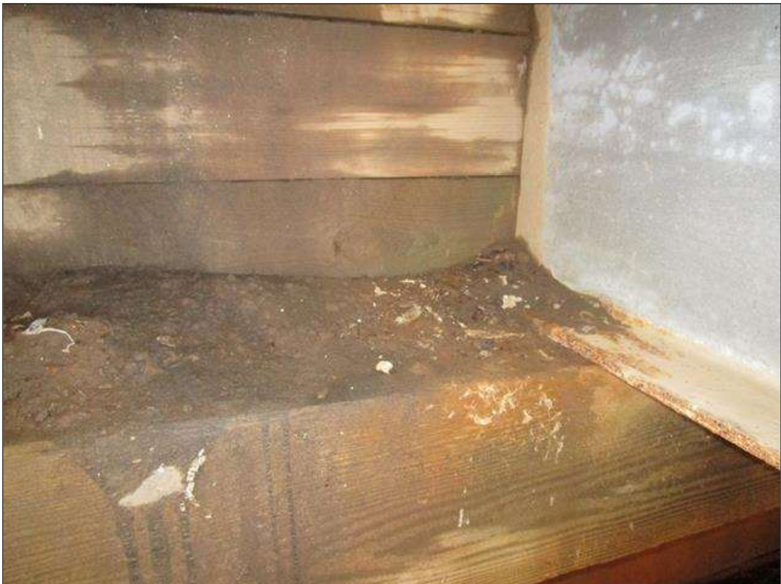
TYPICAL DEBRIS BUILDUP ON END BENT 2 CAP
