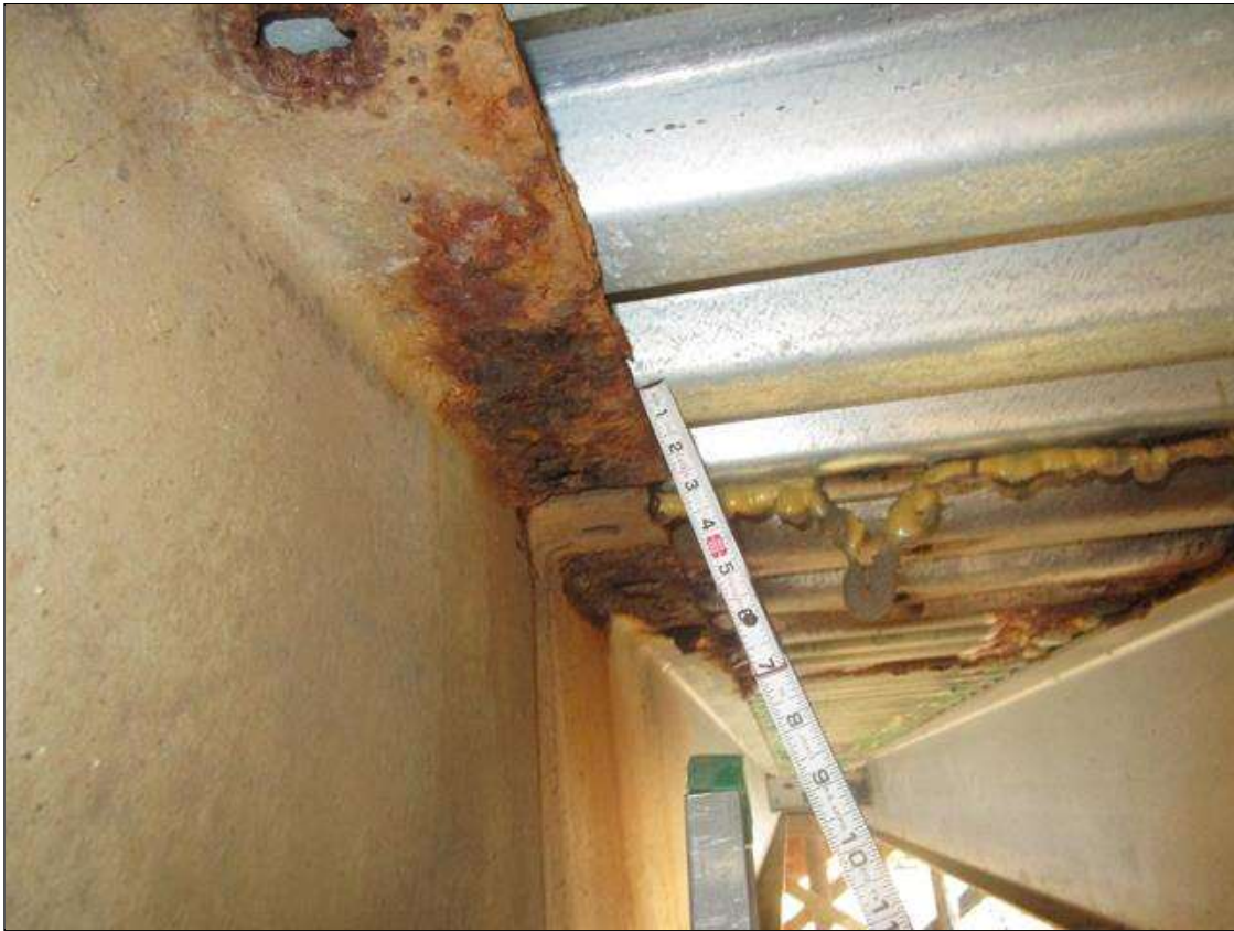
BEAMS 2-7 OVER BENT 1 HAVE CORROSION IN TOP FLANGES. SECTION LOSS IS NEGLIGIBLE AT THIS TIME
