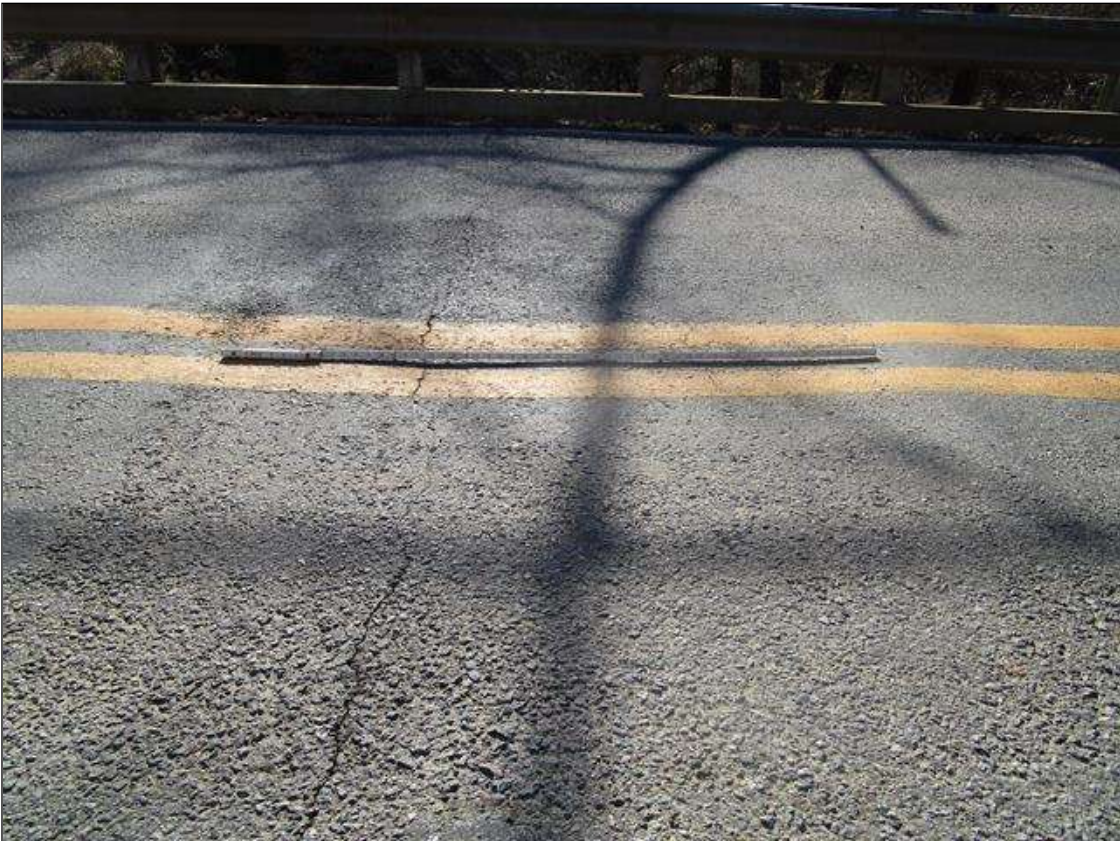
Span 1 Wearing Surface: 6' X 4' AREA OF SUNKEN ASPHALT WEARING SURFACE OVER BENT 1
