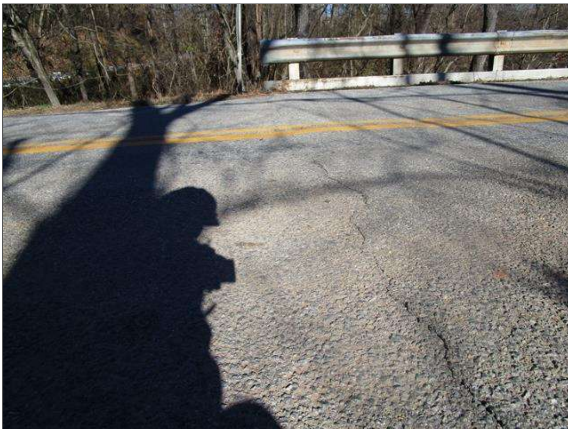
UP TO 1/4" CRACKING AND 1.5" SETTLEMENT IN WEST APPROACH (SIMILAR CONDITIONS AT EAST APPROACH)
