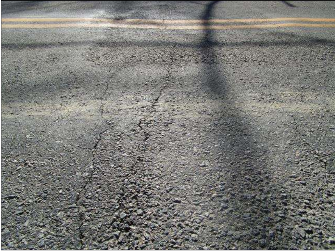
UP TO 1/8" TRANSVERSE CRACKING IN ASPHALT WEARING SURFACE OVER BOTH INTERIOR BENTS
