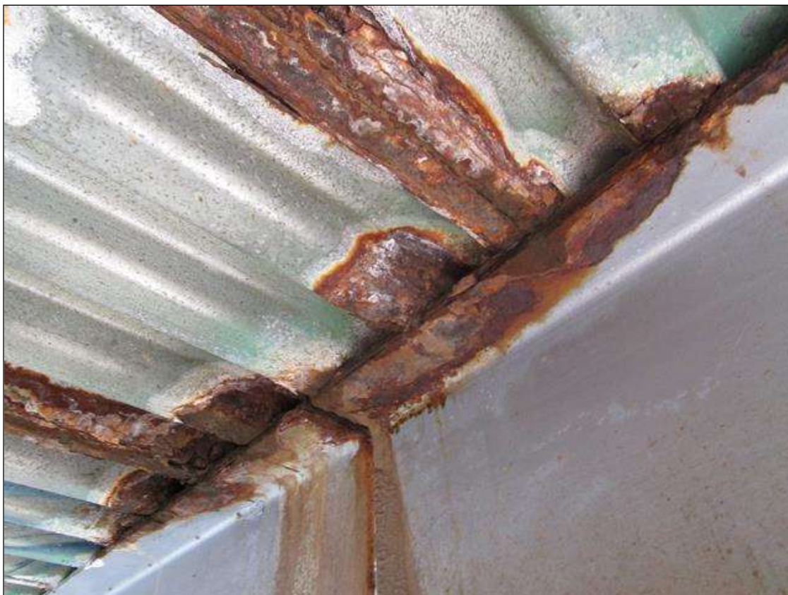
BEAMS 4-8 OVER BENT 2 HAVE CORROSION IN THE TOP FLANGES. SECTION LOSS IS NEGLIGIBLE AT THIS TIME
