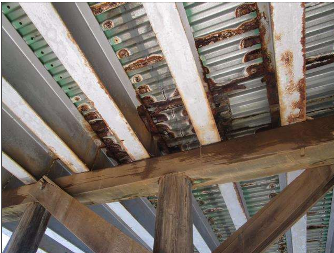
OVERVIEW OF CORROSION TO TOP FLANGES OF BEAMS 4-8 OVER BENT 2
