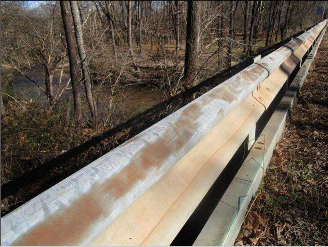
SURFACE RUST ON BOTH RAILS
