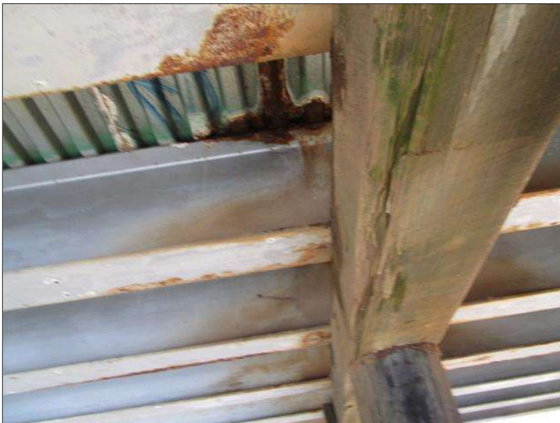
Bent 2 Cap 1: 4 FT X 3 IN WIDE X 2 IN DEEP DELAMINATION IN BOTTOM OF PILE CAP BETWEEN PILES 3 AND 4.
