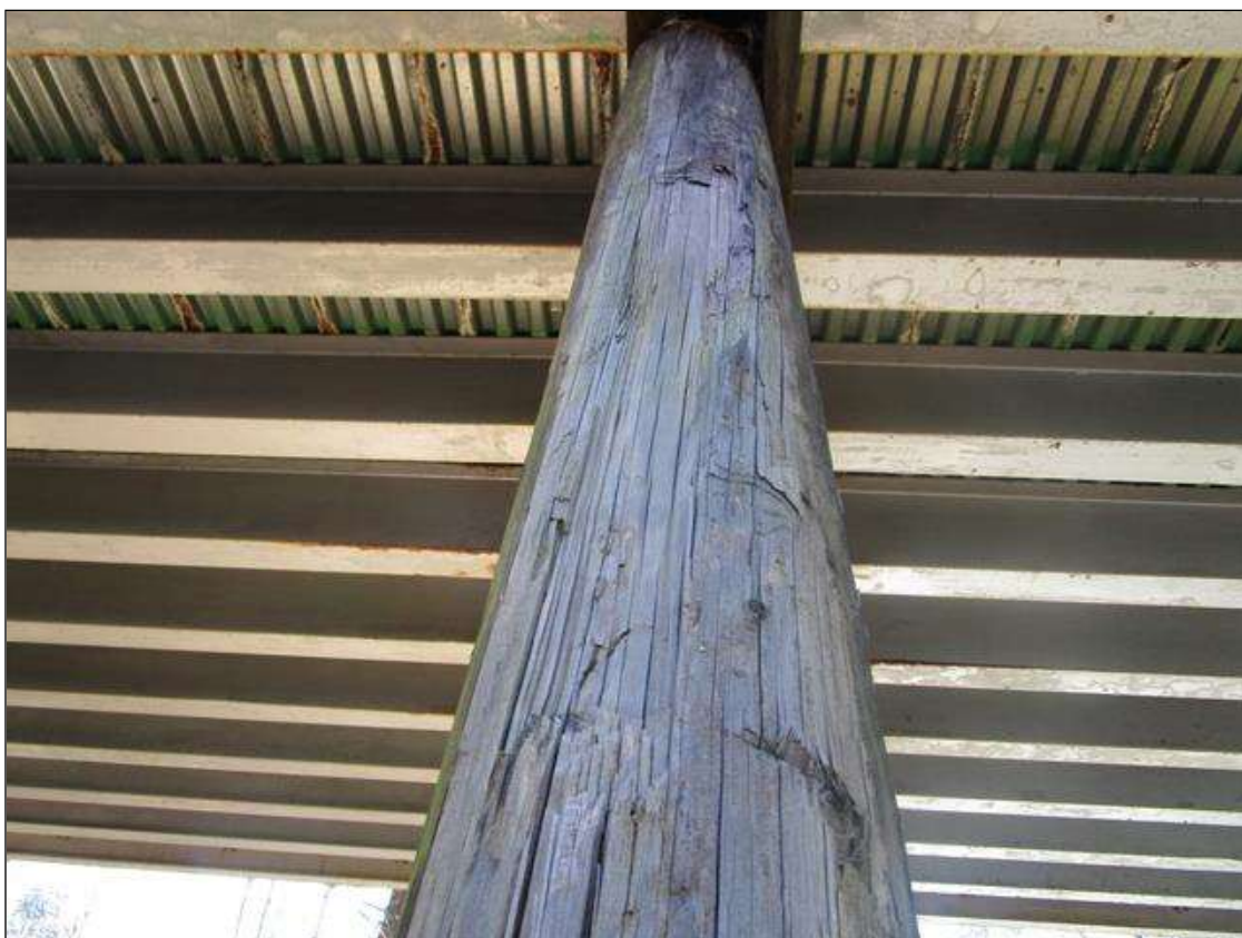
Bent 2 Pile 1: 3 FT HIGH X 6 IN WIDE DELAMINATION, NORTH FACE OF PILE NEAR BASE.
