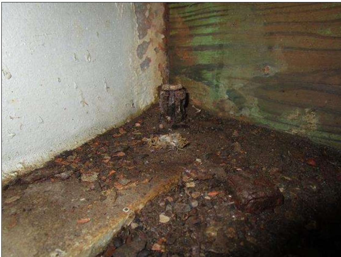
Span 1 Beam 4 Near Bearing: CORROSION OF ANCHOR BOLTS AT END BENT 1, ANCHOR BOLTS MISSING NUTS.
