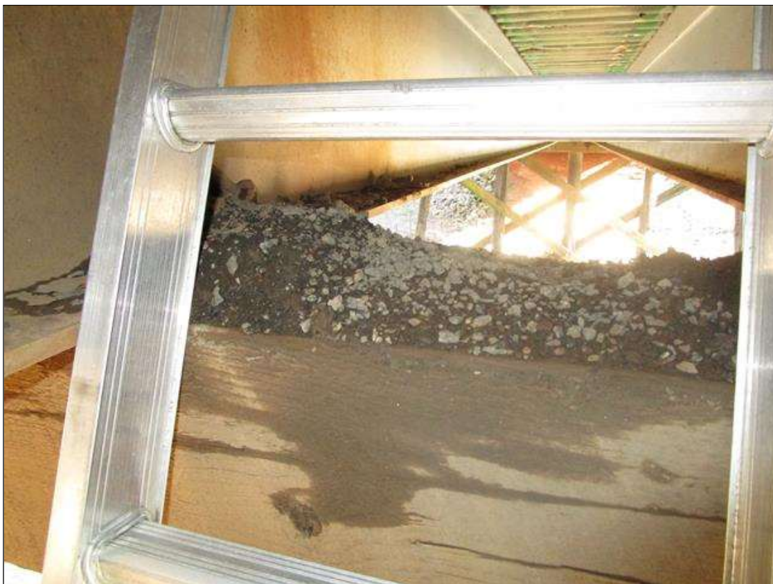
DEBRIS BUILDUP ON BENT 1 CAP
