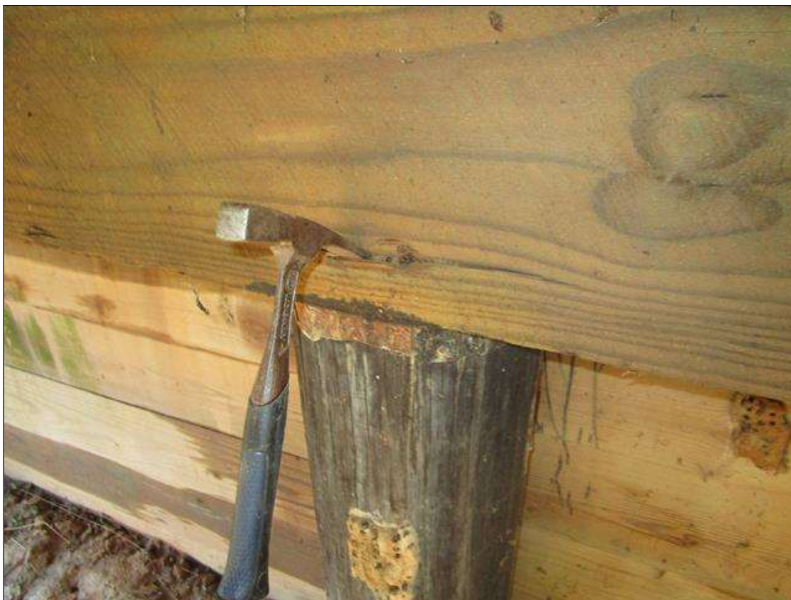
End Bent 1 Cap 1: 1 FT HORIZONTAL SPLIT UP TO 1/8 IN, EAST FACE OF PILE CAP ABOVE PILE 4.
