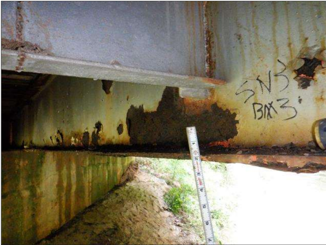
Span 3 Beam 3: [PAR] at midspan, active corrosion with section loss; bottom flange [up to 10ft x full width - avg rem 0.36in], lower web [up to 10ft x 4in - avg rem 5/16in]
