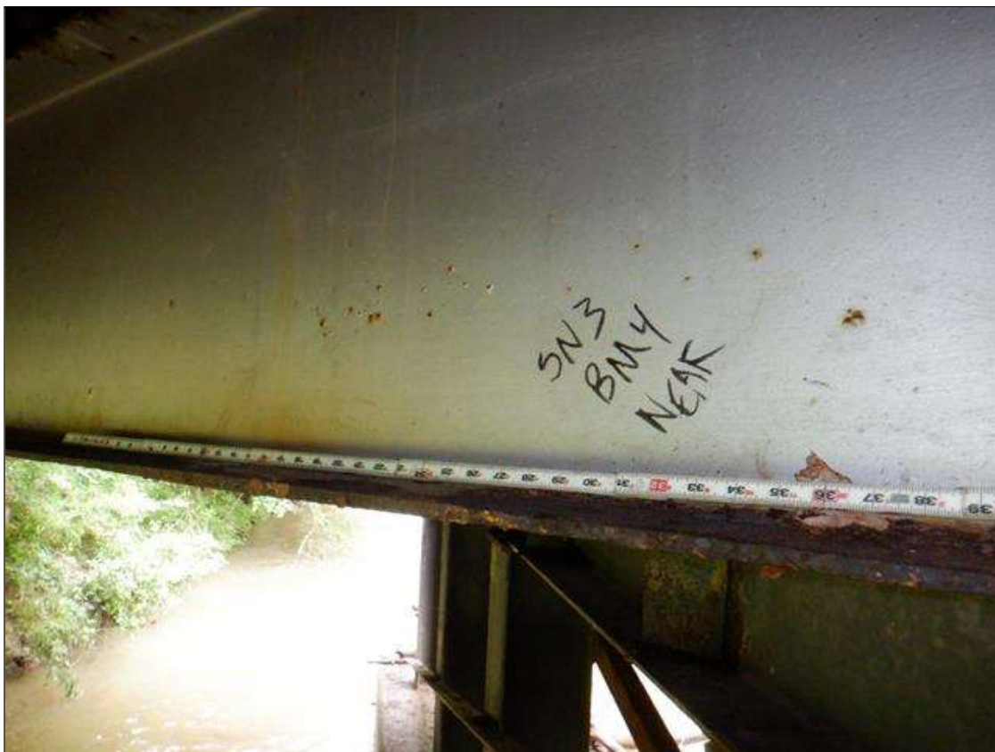
Span 3 Beam 4: [PAR] at near end, active corrosion with section loss; North bottom flange [4ft x 4in - avg rem 3/8in]
