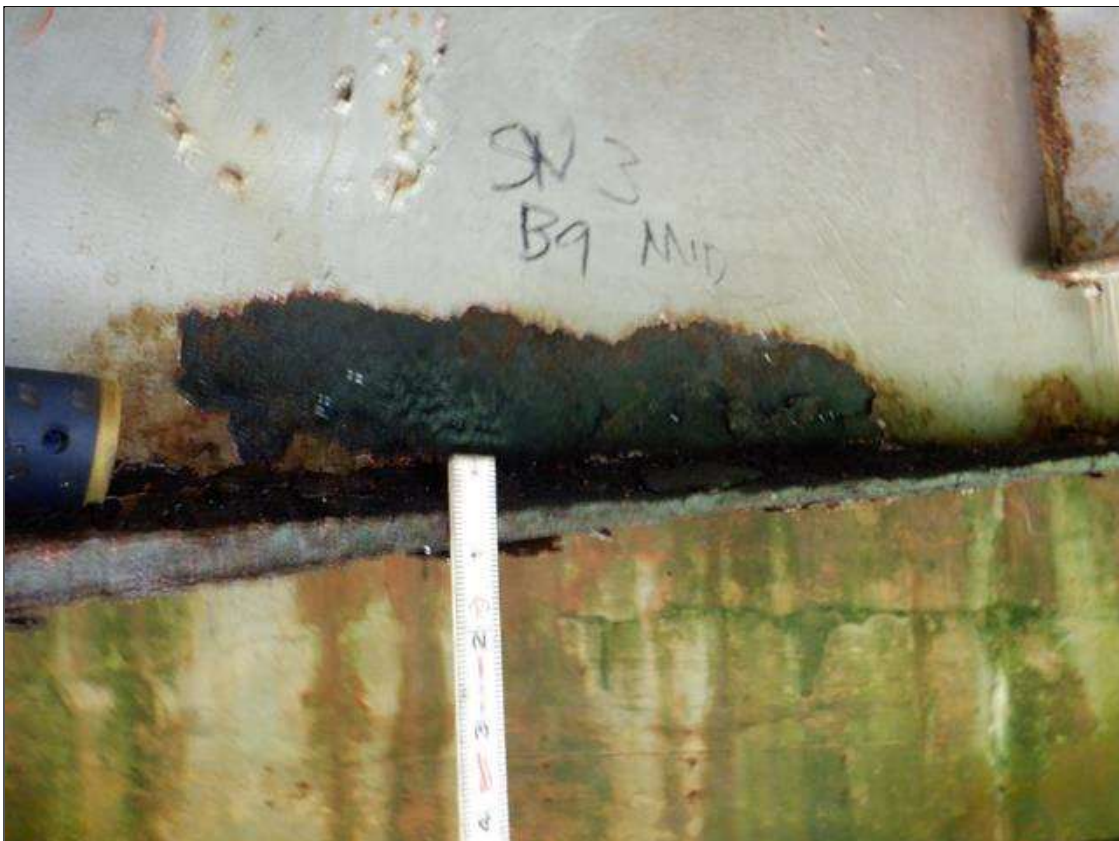
Span 3 Beam 9: [PAR] near midspan, active corrosion with section loss; bottom flange [24in x full width - avg rem 3/8in], lower web [20in x 2in - avg rem 1/4in]
