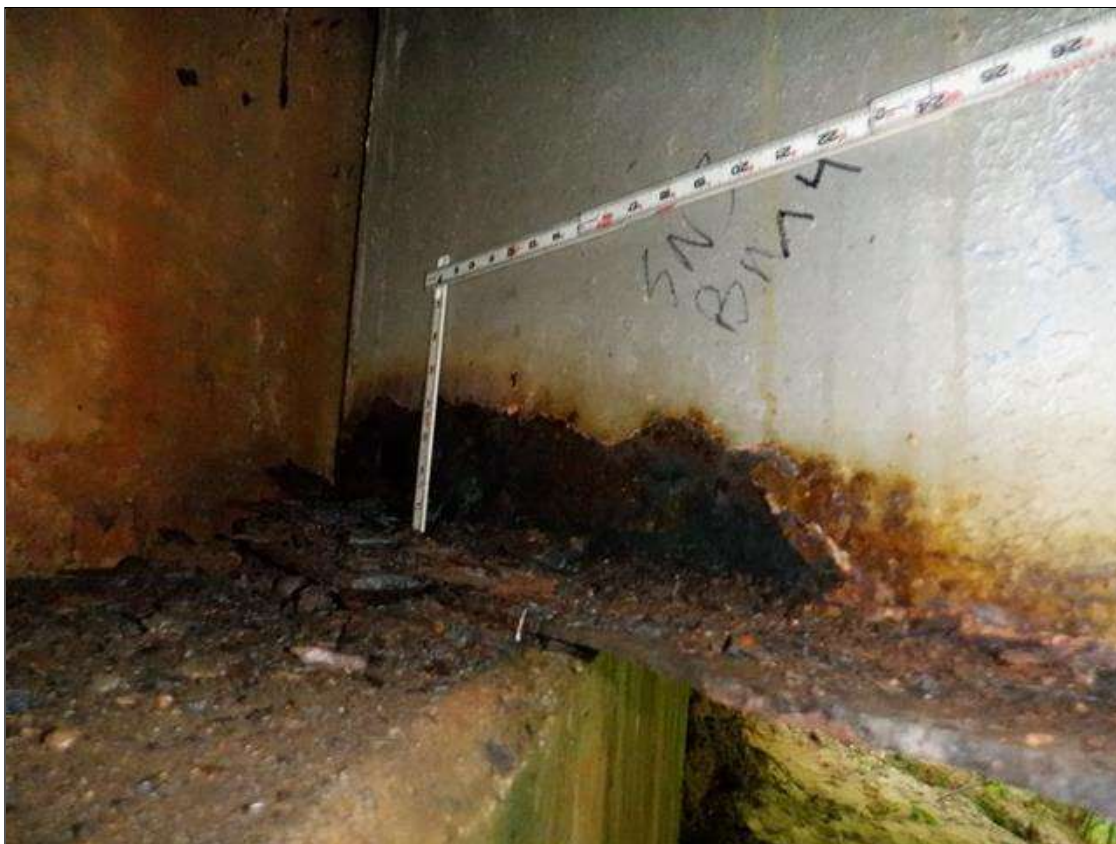
Span 3 Beam 4: [PAR] at far end, active corrosion with section loss, bottom flange [up to 24in x full width - avg rem 3/8in, with areas down to 3/16in], lower web [22in x up to 4in - avg rem 1/4in]
