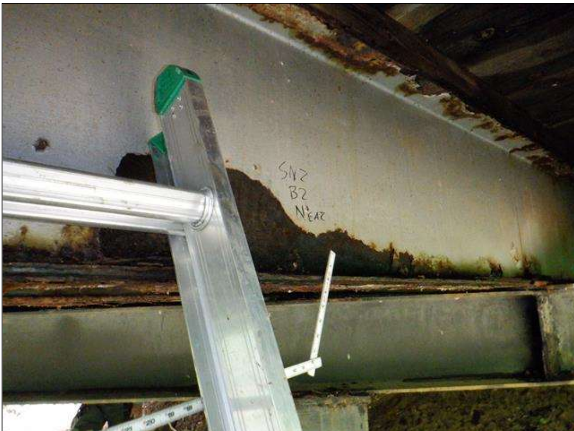
Span 2 Beam 2: [PAR] at near end, active corrosion with section loss; top and bottom flange [12ft x up to full width - avg rem 3/8in], lower web [up to 50in x up to 8in - avg rem 5/16in]
