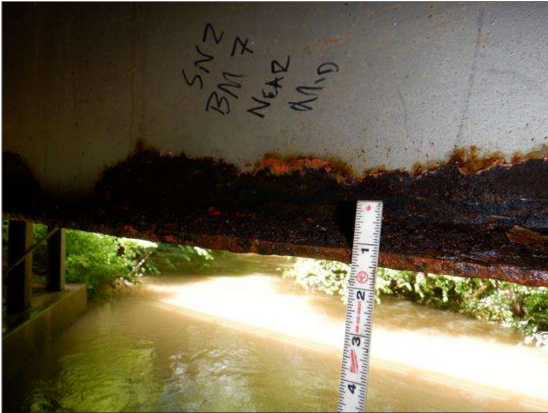
Span 2 Beam 7: [PAR] near midspan, active corrosion with section loss; bottom flange [up to 6ft x full width - avg rem 0.31in], lower web [up to 5ft x 2in - avg rem 5/16in]
