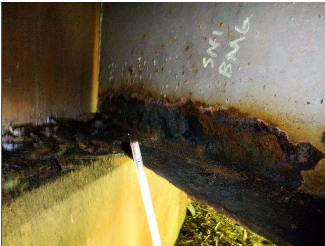
Span 1 Beam 6: [PAR] at near end, active corrosion with section loss, South bottom flange [up to 36in x up to 4in - avg rem 3/8in], lower web [30in x up to 3in - avg rem 1/4in]
