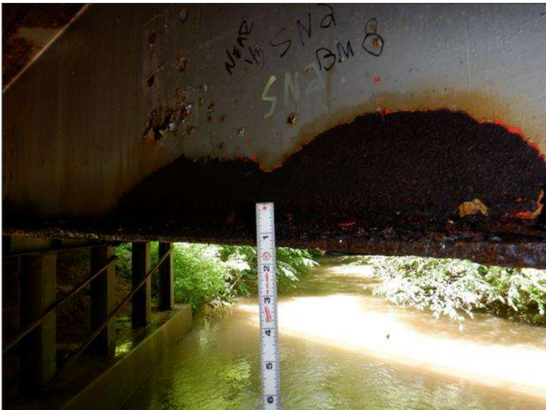
Span 2 Beam 8: [PAR] near midspan, active corrosion with section loss; top and bottom flange [63in x full width - avg rem 3/8in], lower web along length [up to 59in x up to 4in - avg rem 1/4in]
