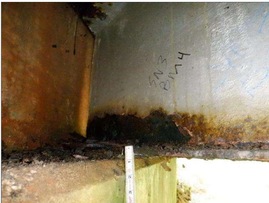
Span 3 Beam 4: [PAR] at far end, active corrosion with section loss, bottom flange [up to 24in x full width - avg rem 3/8in, with areas down to 3/16in], lower web [22in x up to 4in - avg rem 1/4in]
