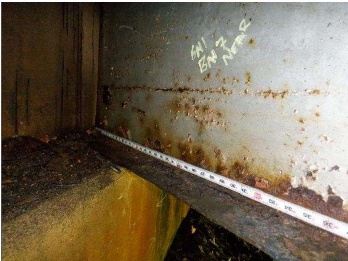
Span 1 Beam 7: [PAR] bottom flange at near end, active corrosion with section loss [up to 30in x up to full width - avg rem 3/8in, with areas down to 1/4in at edges]
