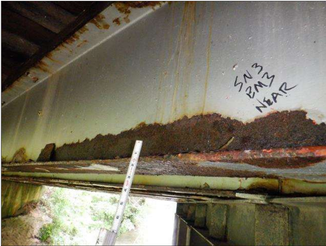
Span 3 Beam 3: [PAR] at 15in from near end, active corrosion with section loss; bottom flange [5ft x up to full width - avg rem 3/8in], lower web [52in x 3in - avg rem 5/16in]
