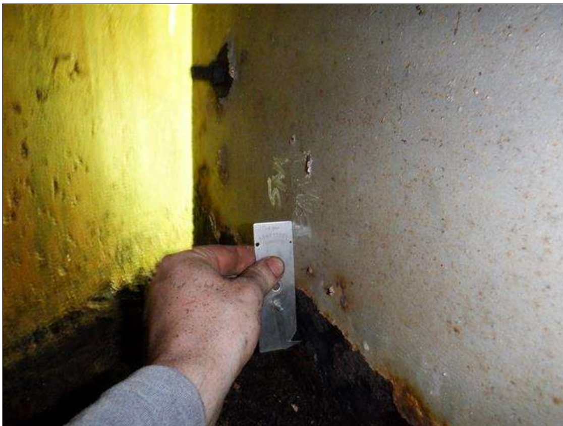
Span 1 Beam 1: [PAR] along length, active corrosion with section loss; top and bottom flange [full length x up to full width - avg rem 1/4in], lower web [full length x up to 3in - avg rem 5/16in]
