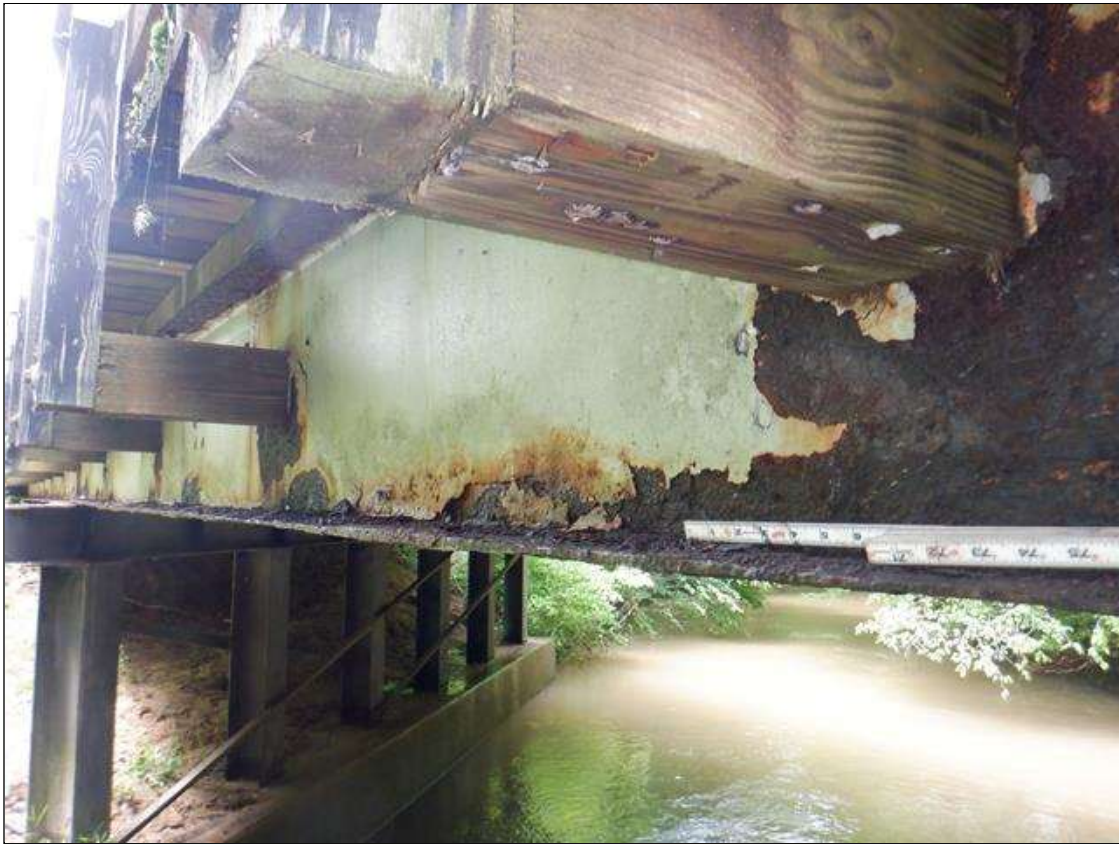
Span 2 Beam 10: [PAR] along length, active corrosion with section loss; top and bottom flange [full length x full width - avg rem 0.34, with areas down to 1/8in], lower web & web at rail connections [up to 3ft x up to 14in - avg rem 1/4in]
