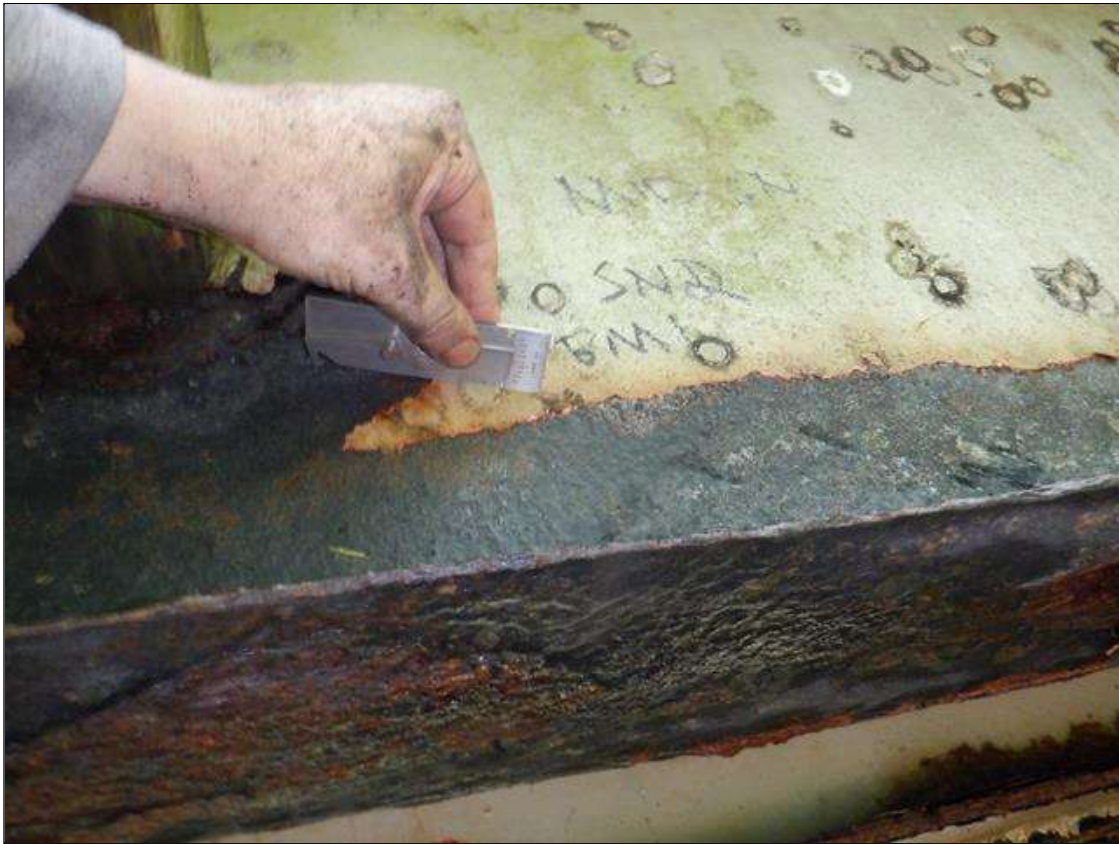
Span 2 Beam 1: [PAR] along length active corrosion with section loss; top and bottom flange [up to 15ft x full width - avg rem 3/8in], bottom flange at midspan [10ft x full width - avg rem 1/4in, with edges down to 1/8in], lower web along length [up to 15ft x up to 9in - avg rem 1/4in], lower web at midspan [10ft x 4in - avg rem 3/16in], web at rail connections [up to 12in diameter - avg rem 1/4in]
