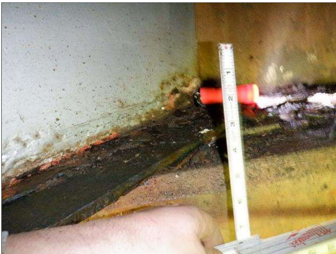
Span 1 Beam 6 Near Bearing: [PAR] North anchor bolt missing
