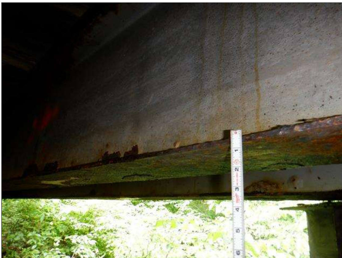
Span 1 Beam 2: [PAR] along length, active corrosion with section loss; top and bottom flange [full length x up to full width - avg rem 0.35in], lower web [up to 3ft x up to 6in - avg rem 5/16in]
