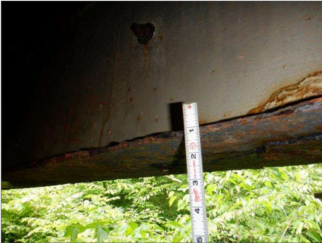
Span 1 Beam 1: [PAR] along length, active corrosion with section loss; top and bottom flange [full length x up to full width - avg rem 1/4in], lower web [full length x up to 3in - avg rem 5/16in]
