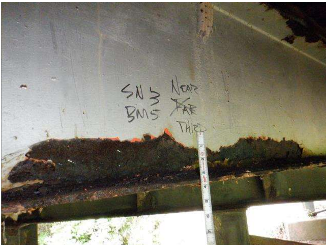
Span 3 Beam 5: [PAR] at near third, active corrosion with section loss; bottom flange [36in x up to full width - avg rem 3/8in], lower web [40in x up to 3in - avg rem 1/4in]
