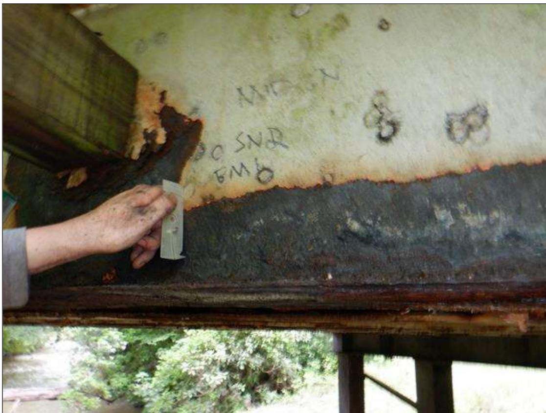
Span 2 Beam 1: [PAR] along length active corrosion with section loss; top and bottom flange [up to 15ft x full width - avg rem 3/8in], bottom flange at midspan [10ft x full width - avg rem 1/4in, with edges down to 1/8in], lower web along length [up to 15ft x up to 9in - avg rem 1/4in], lower web at midspan [10ft x 4in - avg rem 3/16in], web at rail connections [up to 12in diameter - avg rem 1/4in]
