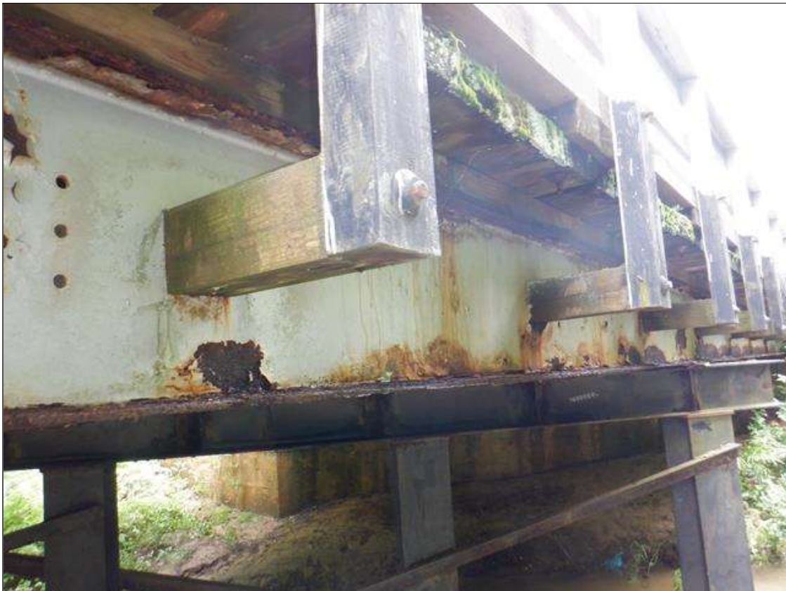
Span 2 Beam 10: [PAR] along length, active corrosion with section loss; top and bottom flange [full length x full width - avg rem 0.34, with areas down to 1/8in], lower web & web at rail connections [up to 3ft x up to 14in - avg rem 1/4in]
