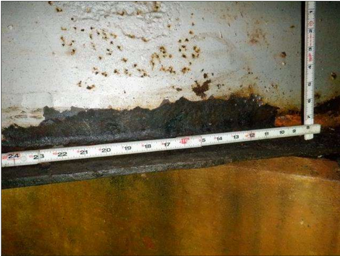
Span 1 Beam 8: [PAR] at near end, active corrosion with section loss; bottom flange [22in x full width - avg rem 1/4in], lower web [28in x up to 2-1/2in - avg rem 1/4in]
