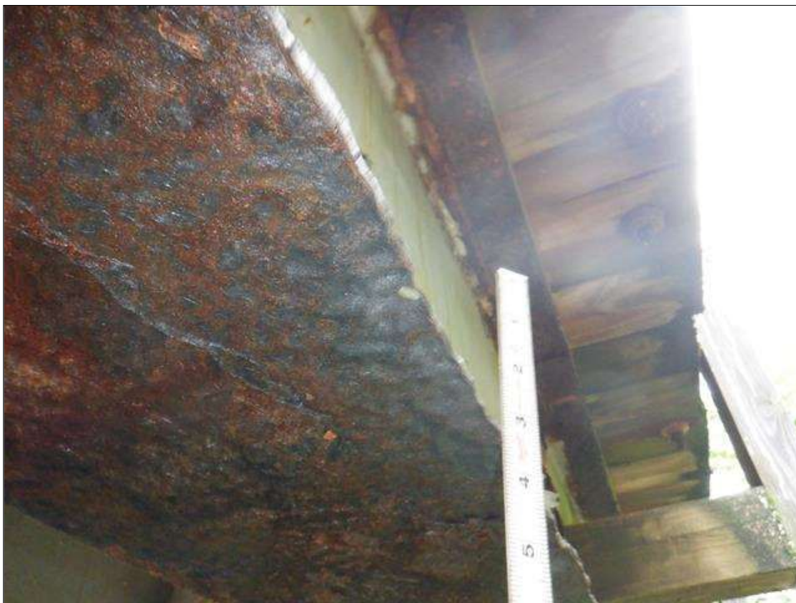
Span 3 Beam 10: [PAR] along length, active corrosion with section loss; top and bottom flange [full length x up to full width - avg rem 1/4in, with edges down to 1/16in], lower web [full length x up to 4in - avg rem 1/4in, with areas down to 3/16in], web at rail attachments [12in diameter - avg rem 1/4in]
