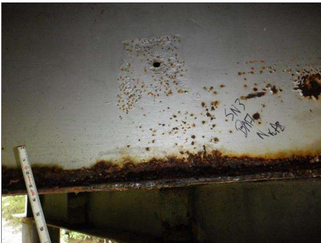
Span 3 Beam 7: [PAR] at 18in from near end, active corrosion with section loss; bottom flange [32in x up to full width - avg rem 3/8in]
