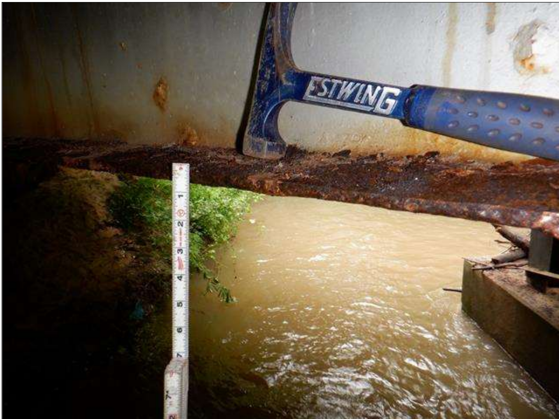
Span 3 Beam 4: [PAR] near midspan, active corrosion with section loss; top flange [up to 30in x up to full width - avg rem 5/16in], bottom flange [62in x up to full width - avg rem 7/16in]
