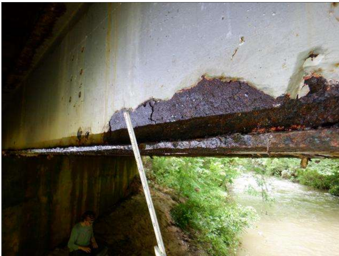
Span 3 Beam 2: [PAR] near midspan, active corrosion with section loss, bottom flange [10ft x full width - avg rem 0.35in], lower web [10ft x 4in - avg rem 5/16in]
