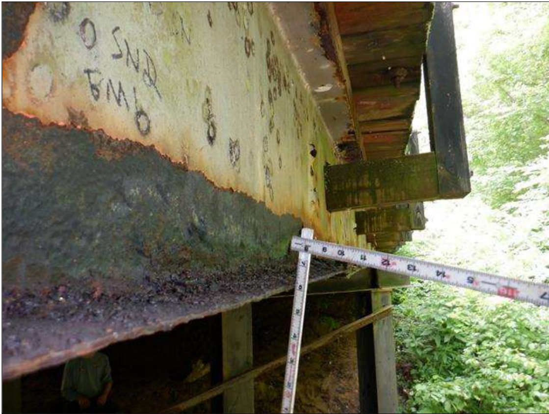
Span 2 Beam 1: [PAR] along length active corrosion with section loss; top and bottom flange [up to 15ft x full width - avg rem 3/8in], bottom flange at midspan [10ft x full width - avg rem 1/4in, with edges down to 1/8in], lower web along length [up to 15ft x up to 9in - avg rem 1/4in], lower web at midspan [10ft x 4in - avg rem 3/16in], web at rail connections [up to 12in diameter - avg rem 1/4in]
