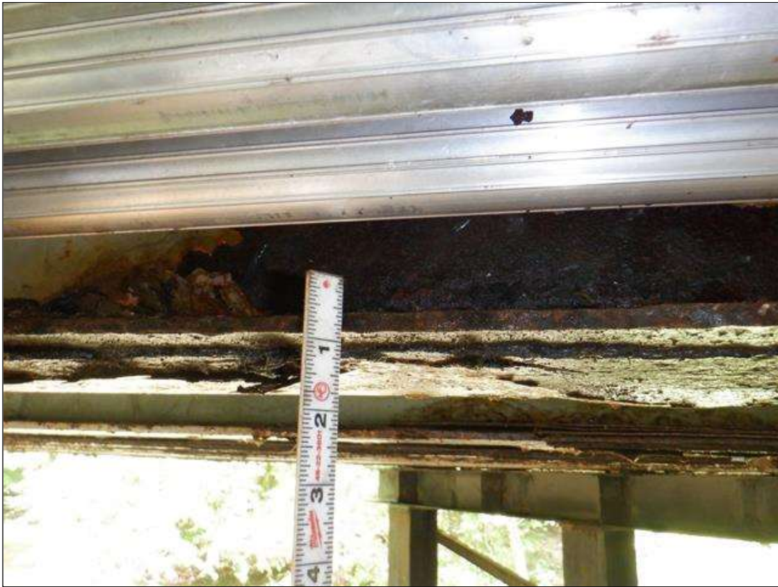
Span 2 Beam 8: [PAR] near midspan, active corrosion with section loss; top and bottom flange [63in x full width - avg rem 3/8in], lower web along length [up to 59in x up to 4in - avg rem 1/4in]
