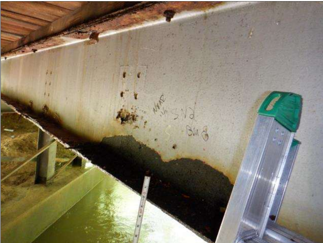
Span 2 Beam 8: [PAR] near midspan, active corrosion with section loss; top and bottom flange [63in x full width - avg rem 3/8in], lower web along length [up to 59in x up to 4in - avg rem 1/4in]
