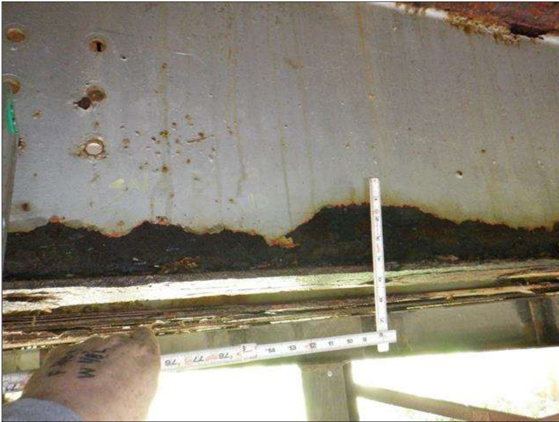
Span 2 Beam 8: [PAR] near midspan, active corrosion with section loss; top and bottom flange [63in x full width - avg rem 3/8in], lower web along length [up to 59in x up to 4in - avg rem 1/4in]
