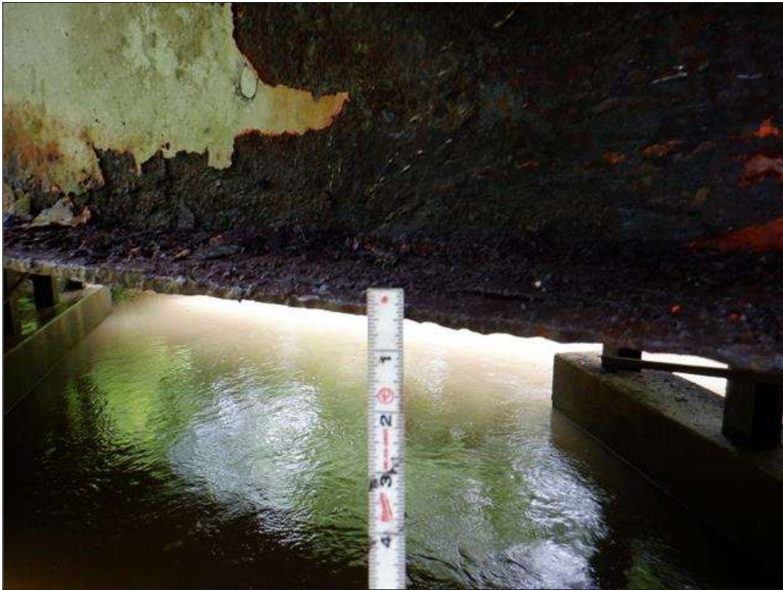
Span 2 Beam 10: [PAR] along length, active corrosion with section loss; top and bottom flange [full length x full width - avg rem 0.34, with areas down to 1/8in], lower web & web at rail connections [up to 3ft x up to 14in - avg rem 1/4in]
