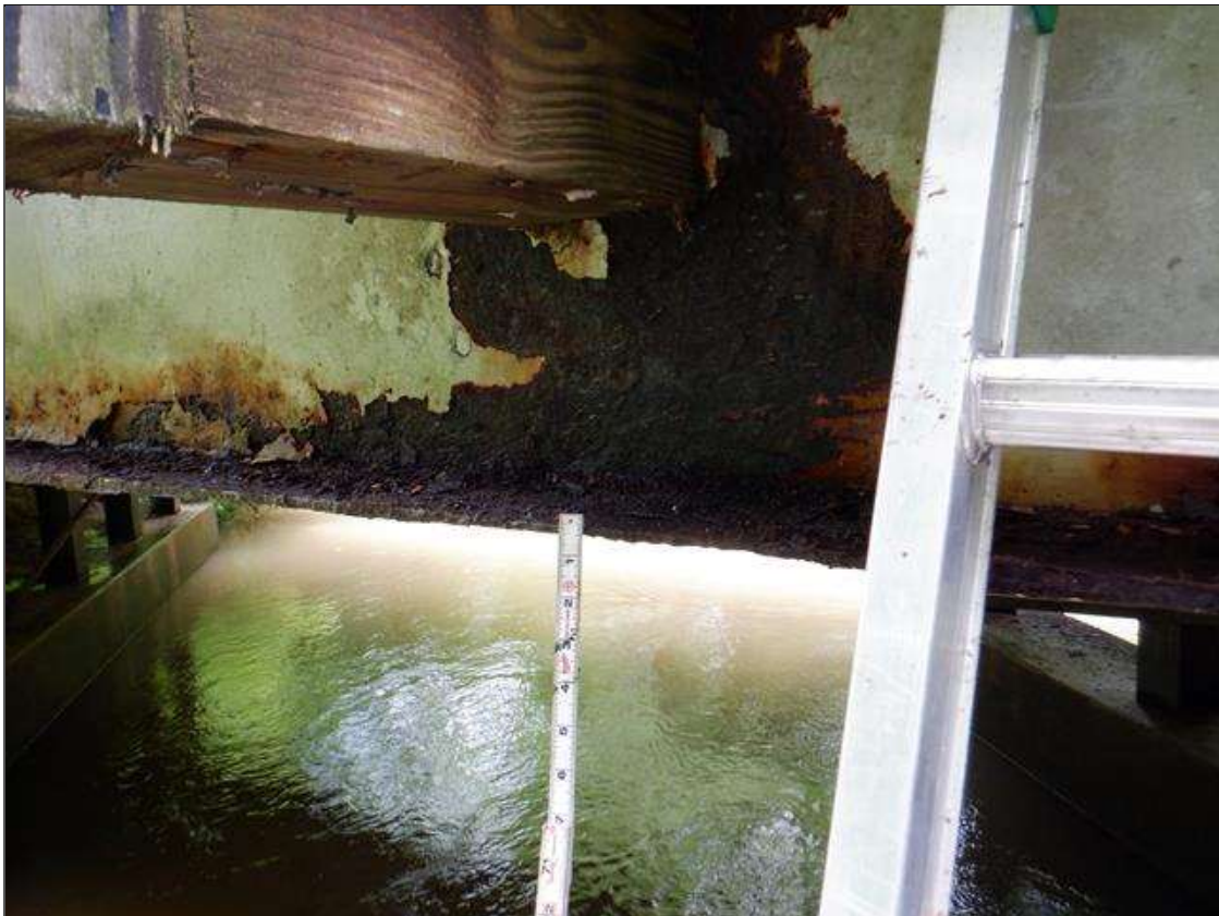
Span 2 Beam 10: [PAR] along length, active corrosion with section loss; top and bottom flange [full length x full width - avg rem 0.34, with areas down to 1/8in], lower web & web at rail connections [up to 3ft x up to 14in - avg rem 1/4in]
