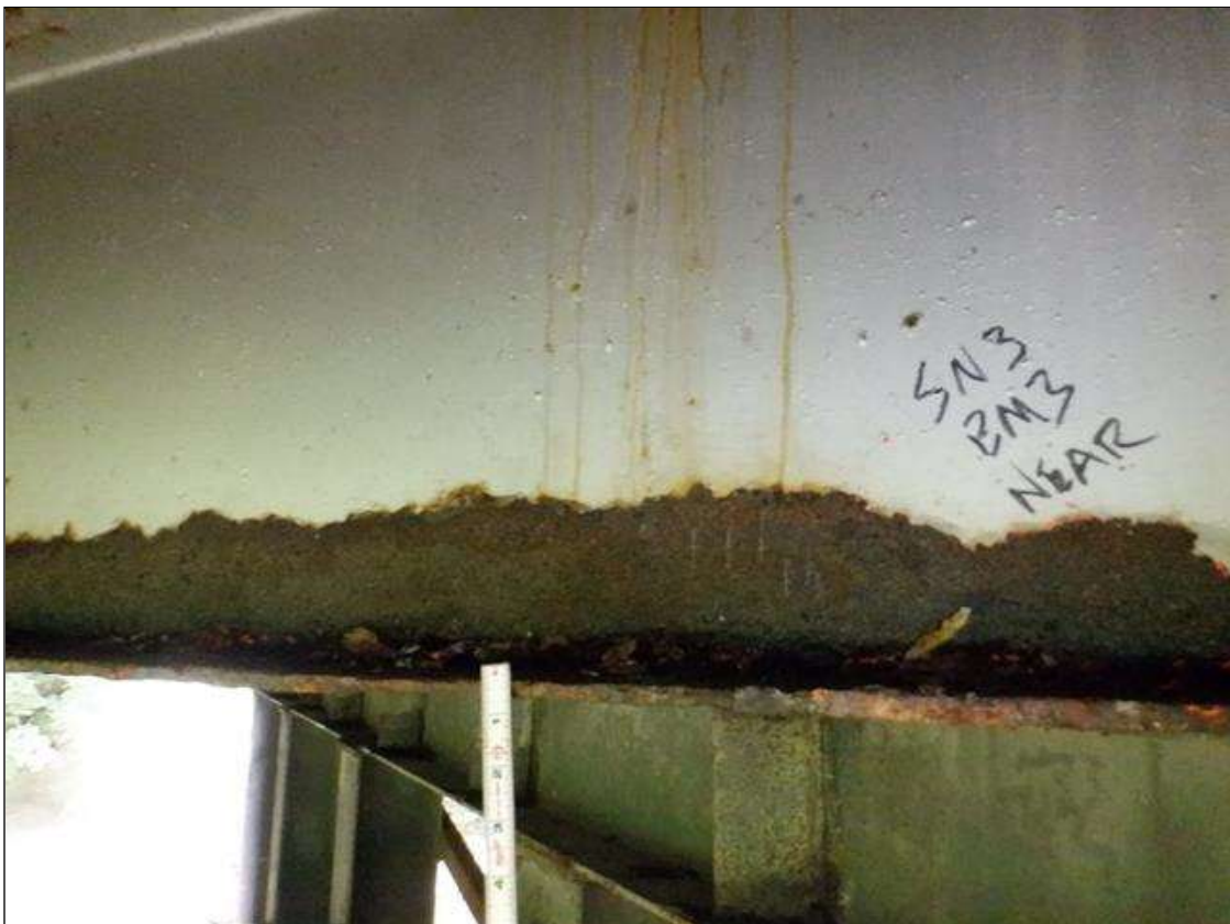
Span 3 Beam 3: [PAR] at 15in from near end, active corrosion with section loss; bottom flange [5ft x up to full width - avg rem 3/8in], lower web [52in x 3in - avg rem 5/16in]
