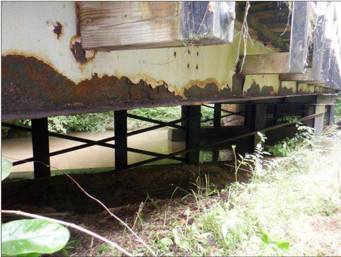
Span 1 Beam 10: [PAR] along length of beam, multiple areas of active corrosion with section loss; bottom flange [up to 68in x 6in - avg rem 1/4in], lower web & web at rail post connections [up to 10ft x 6in - avg rem 1/4in]
