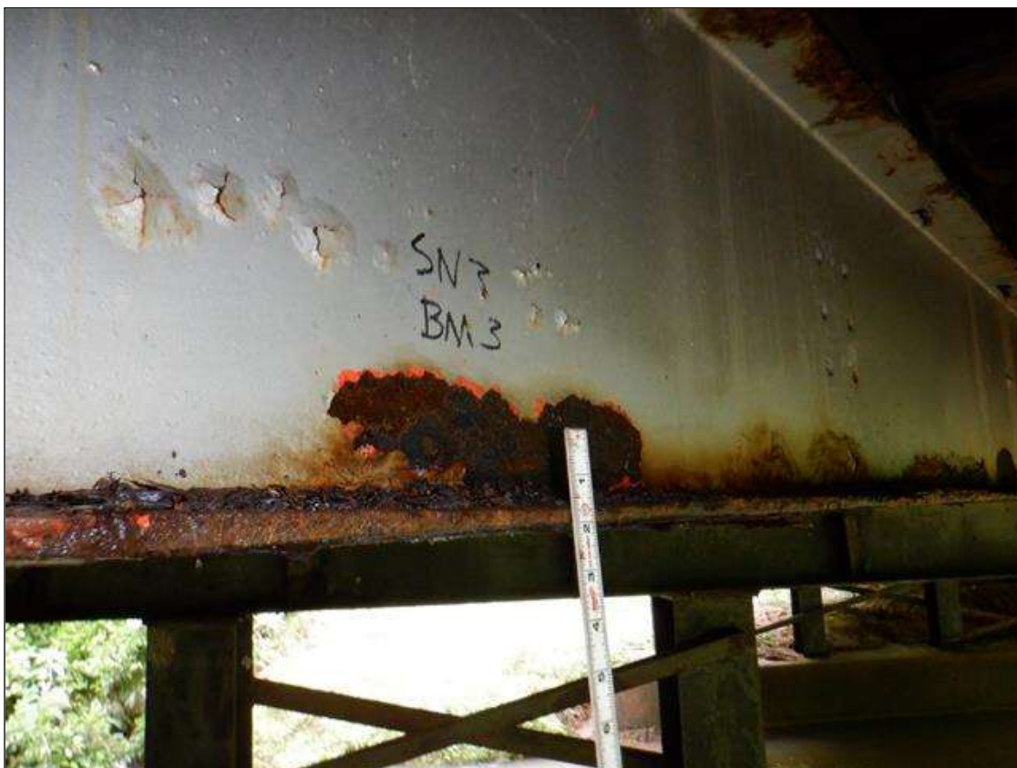
Span 3 Beam 3: [PAR] at midspan, active corrosion with section loss; bottom flange [up to 10ft x full width - avg rem 0.36in], lower web [up to 10ft x 4in - avg rem 5/16in]
