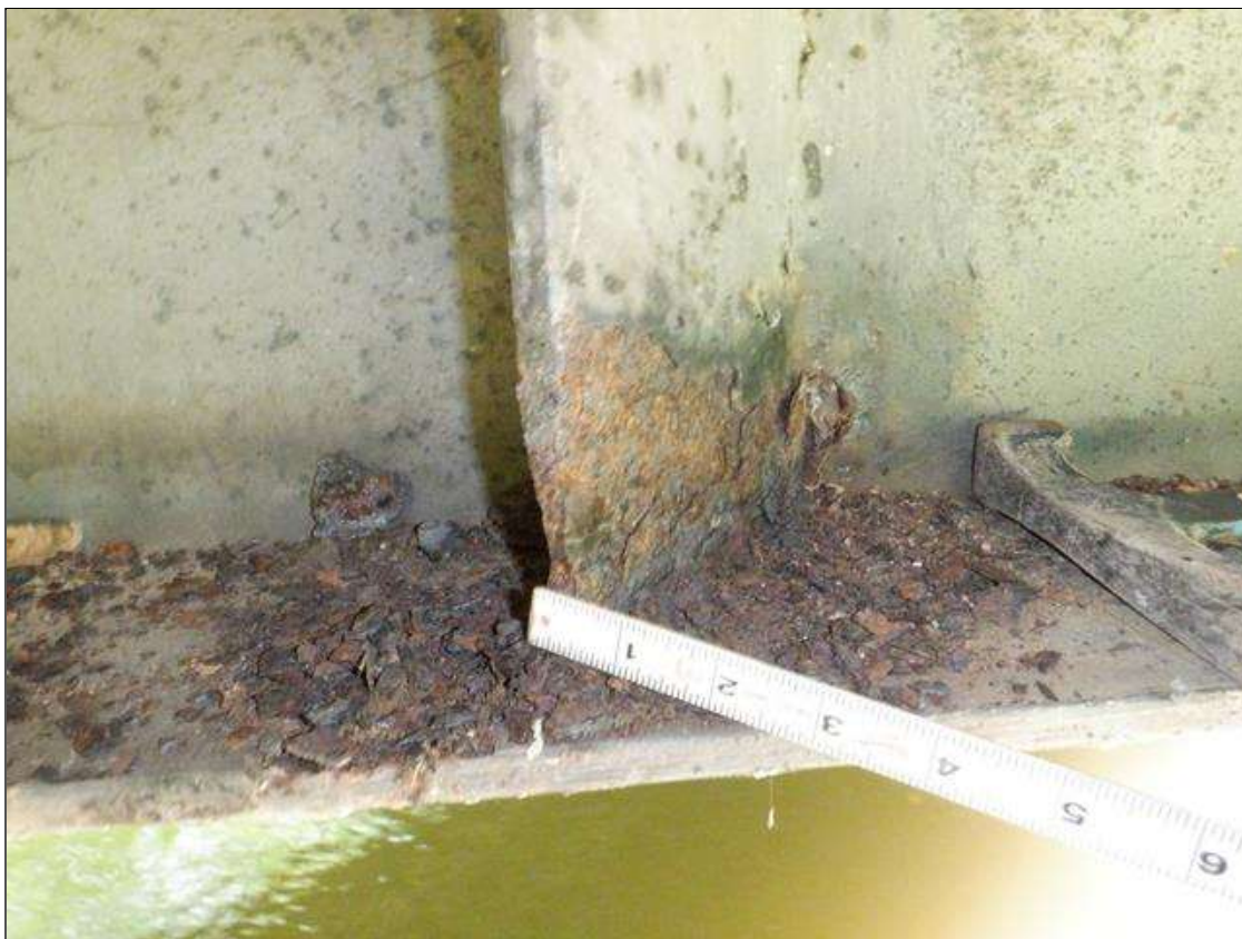
Bent 1 Cap 1: [PAR] along West face at stiffeners 2-6, 9, & 10, active corrosion with section loss [up to 6in x full width - avg rem 3/8in]; along East face at stiffeners 1-5, 9 & 10, active corrosion with section loss [8in x full width - avg rem 3/8in]
