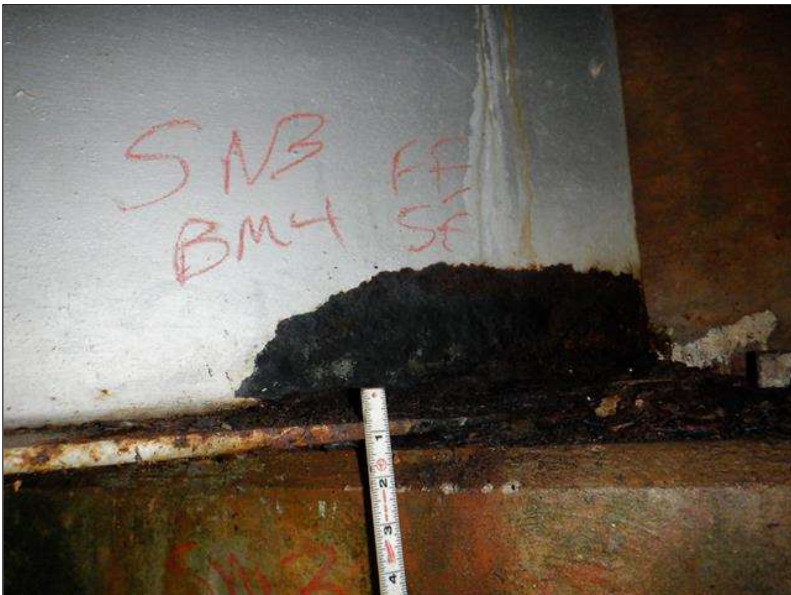
Span 3 Beam 4: [PAR] at far end, active corrosion with section loss, bottom flange [up to 24in x full width - avg rem 3/8in, with areas down to 3/16in], lower web [22in x up to 4in - avg rem 1/4in]
