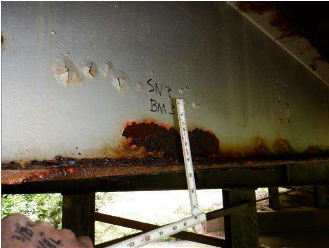
Span 3 Beam 3: [PAR] at midspan, active corrosion with section loss; bottom flange [up to 10ft x full width - avg rem 0.36in], lower web [up to 10ft x 4in - avg rem 5/16in]
