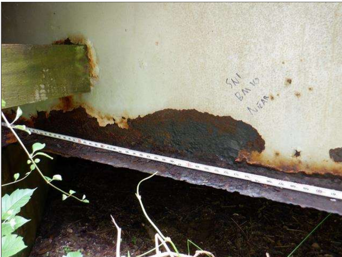
Span 1 Beam 10: [PAR] along length of beam, multiple areas of active corrosion with section loss; bottom flange [up to 68in x 6in - avg rem 1/4in], lower web & web at rail post connections [up to 10ft x 6in - avg rem 1/4in]
