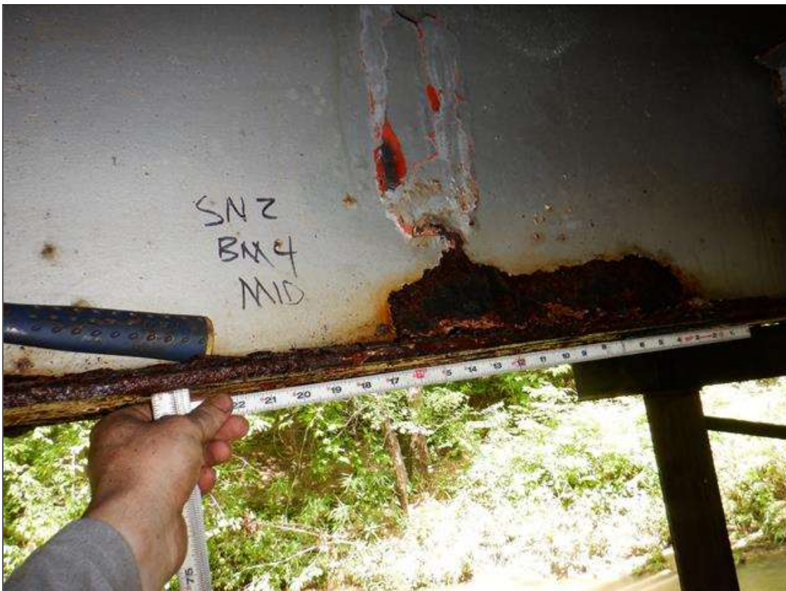
Span 2 Beam 4: [PAR] near midspan, active corrosion with section loss; bottom flange [up to 42in x up to full width - avg rem 3/8in], lower web [16in x 2in - avg rem 1/4in]
