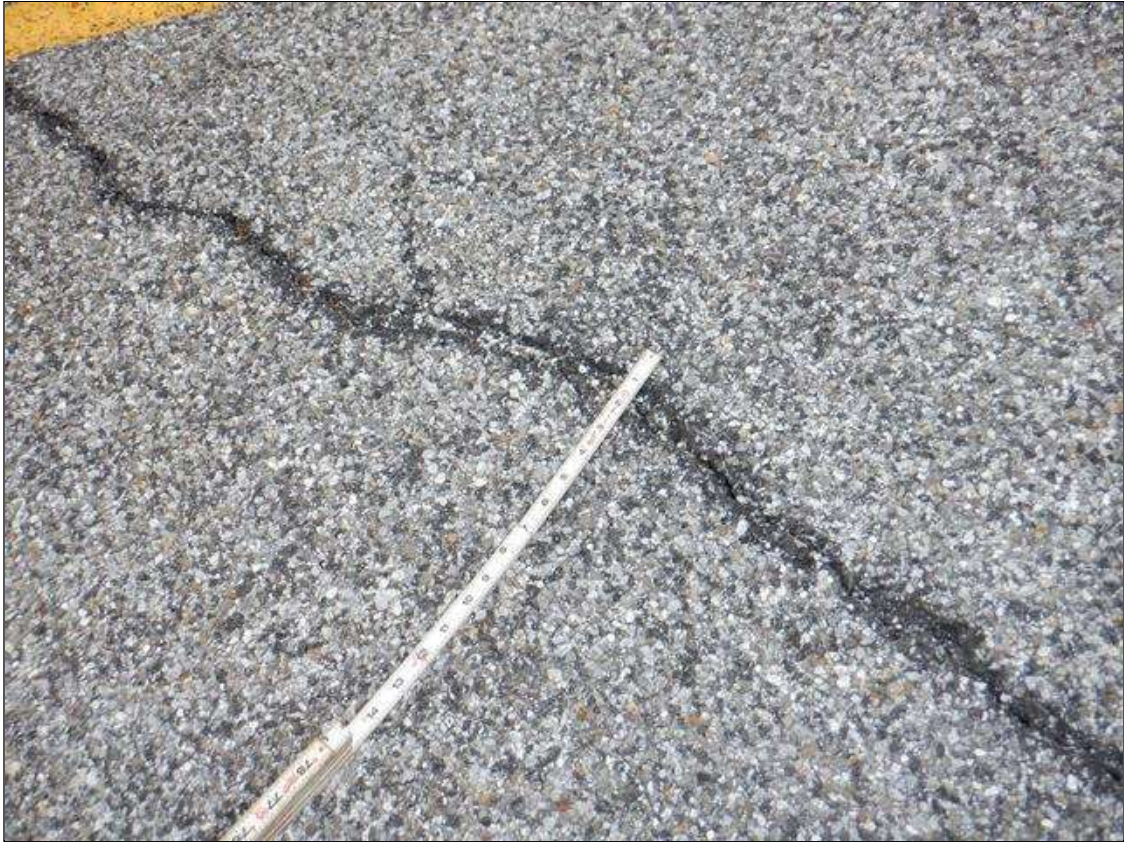
Span 1 Wearing Surface: both lanes and shoulders over end bent 1, transverse crack (full width x up to 1in)
