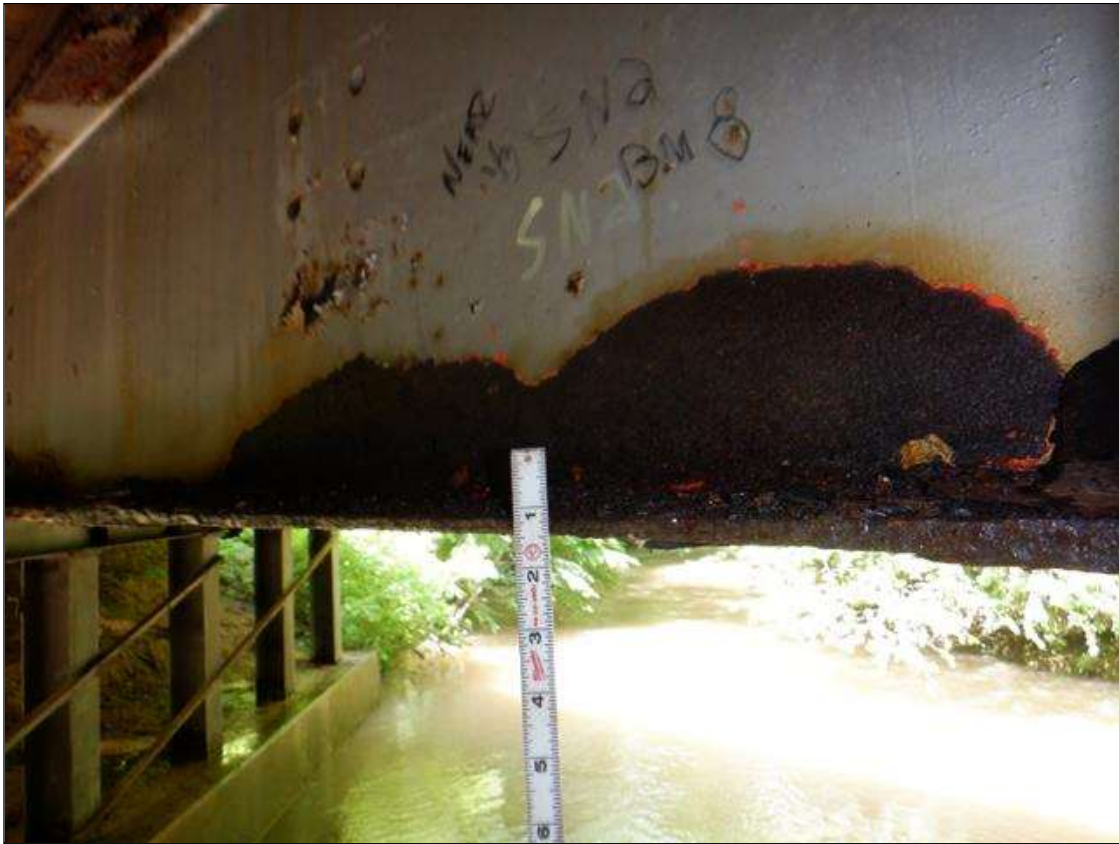
Span 2 Beam 8: [PAR] near midspan, active corrosion with section loss; top and bottom flange [63in x full width - avg rem 3/8in], lower web along length [up to 59in x up to 4in - avg rem 1/4in]
