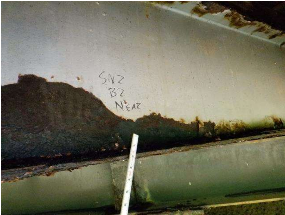
Span 2 Beam 2: [PAR] at near end, active corrosion with section loss; top and bottom flange [12ft x up to full width - avg rem 3/8in], lower web [up to 50in x up to 8in - avg rem 5/16in]
