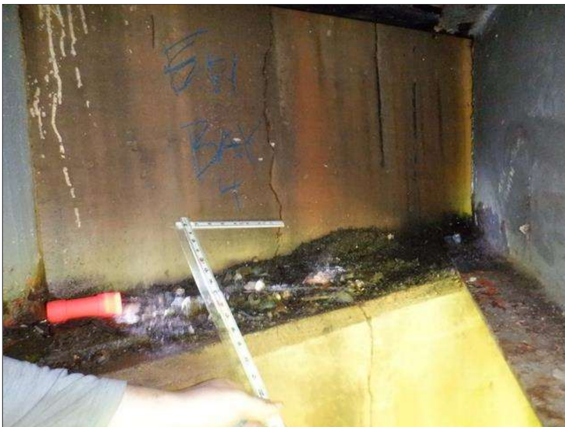
End Bent 1 Abutment/Backwall : at bay 4, vertical crack [full height x 3/16in]
