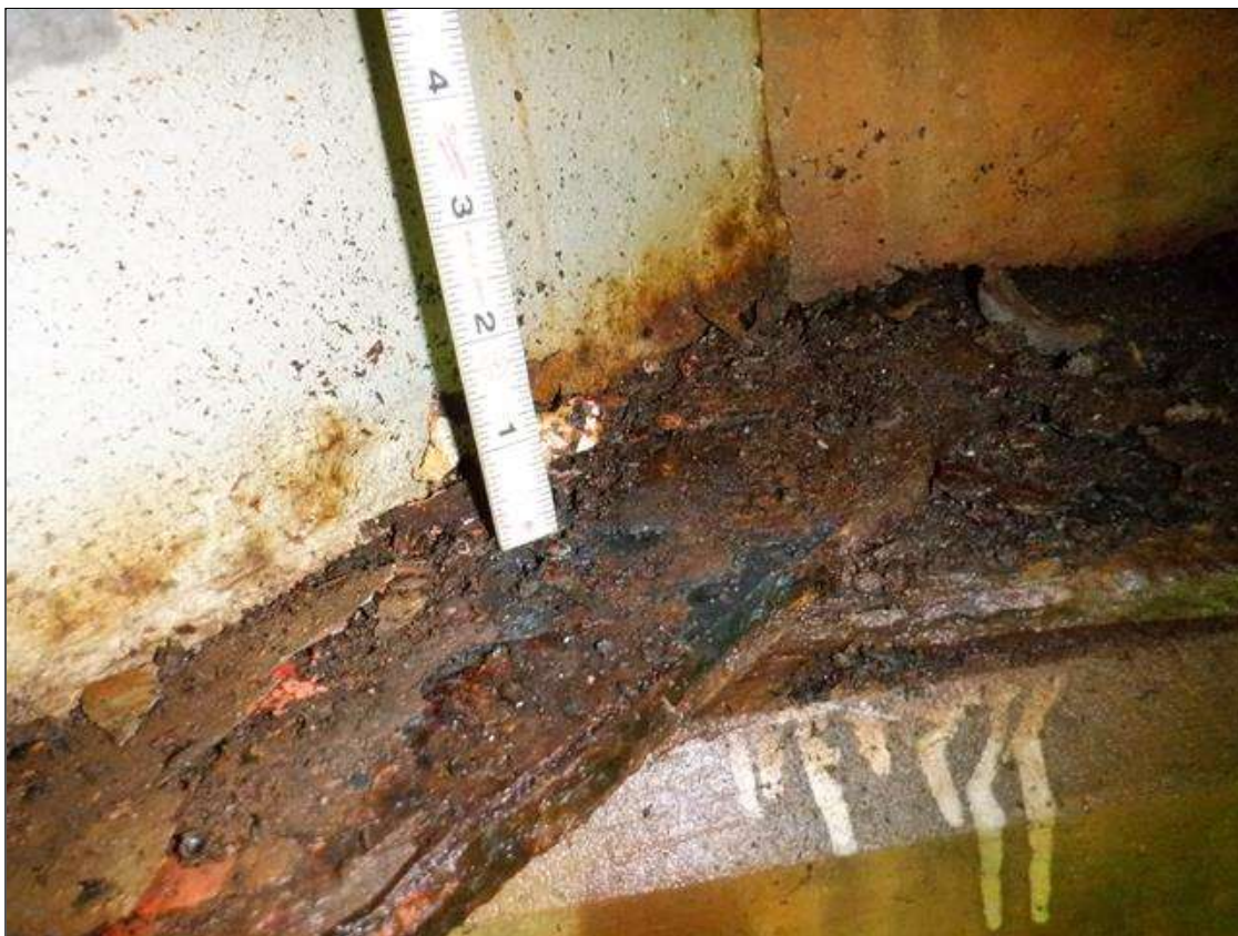
Span 1 Beam 2 Near Bearing: [PAR] North anchor bolt missing
