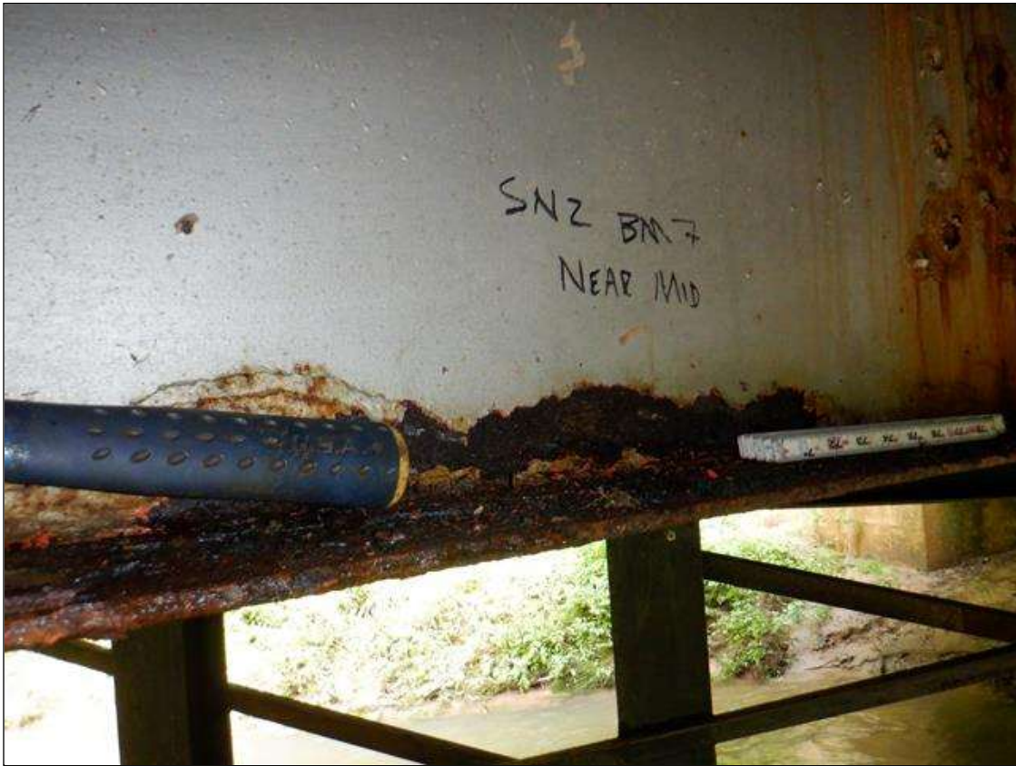
Span 2 Beam 7: [PAR] near midspan, active corrosion with section loss; bottom flange [up to 6ft x full width - avg rem 0.31in], lower web [up to 5ft x 2in - avg rem 5/16in]
