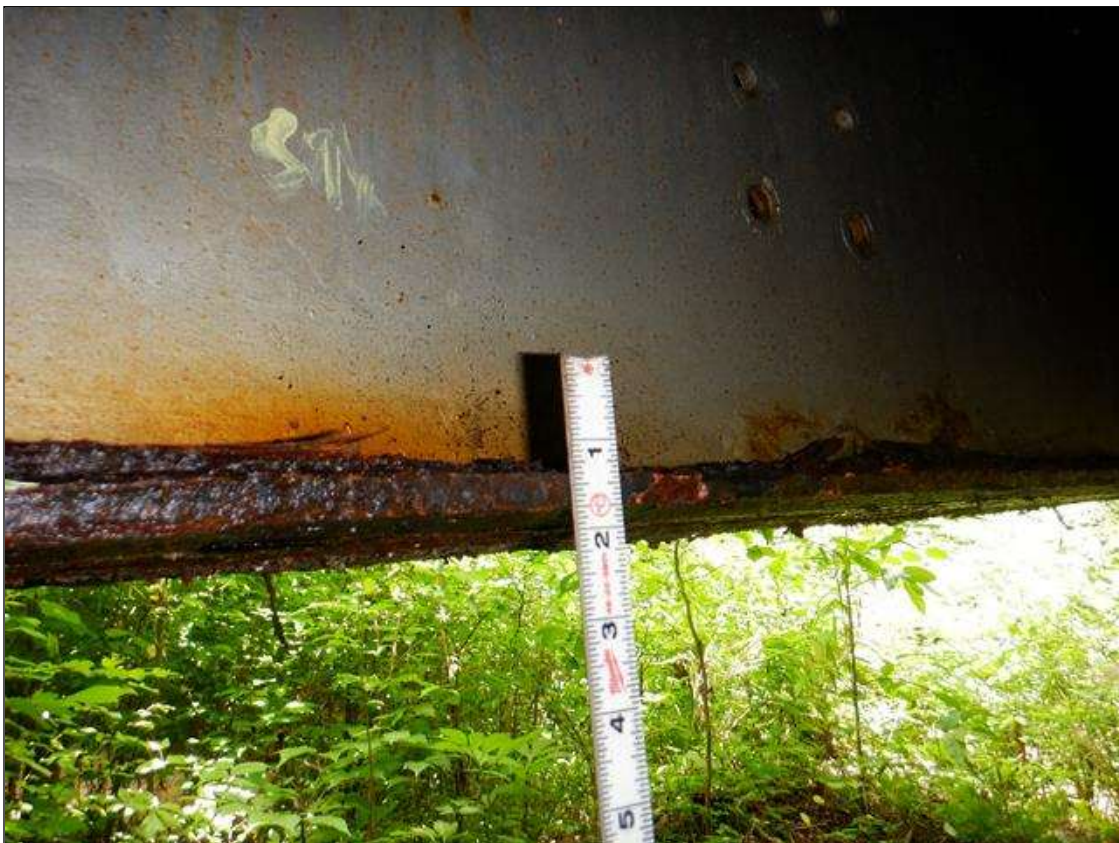
Span 1 Beam 2: [PAR] along length, active corrosion with section loss; top and bottom flange [full length x up to full width - avg rem 0.35in], lower web [up to 3ft x up to 6in - avg rem 5/16in]
