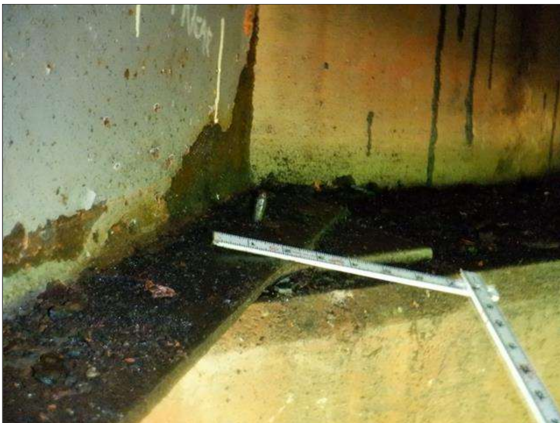
Span 1 Beam 9 Near Bearing: [PAR] North anchor bolt nut missing, [1/8in loss] on bolt and not fully embedded
