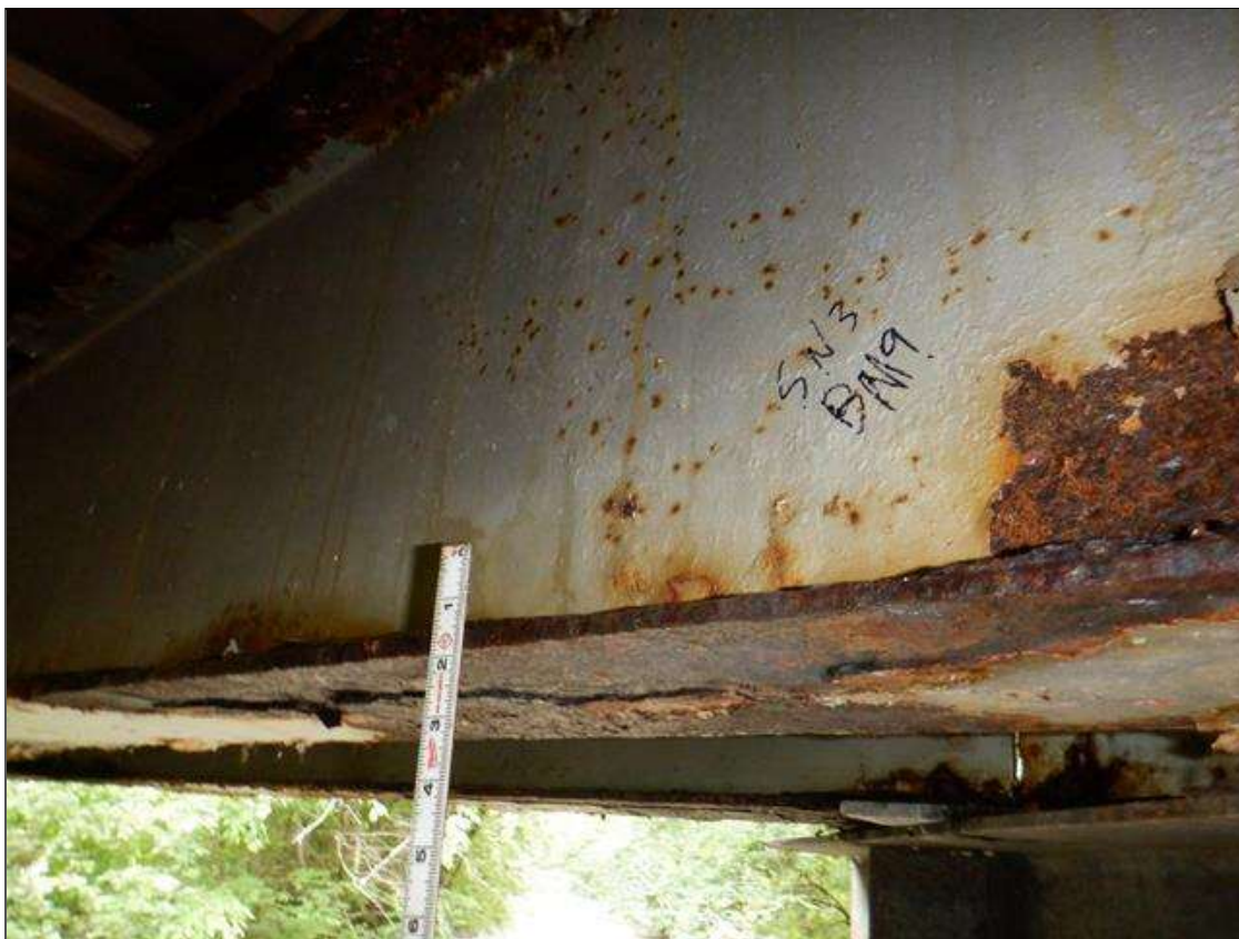
Span 3 Beam 9: [PAR] at near end, active corrosion with section loss; North bottom flange [41in x 4in - avg rem 3/8in]
