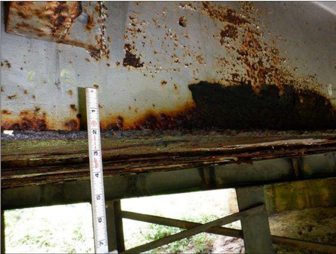
Span 2 Beam 9: [PAR] at midspan, active corrosion with section loss; bottom flange [2ft x full width - avg rem 3/8in], lower web [32in x 5in - avg rem 1/4in]
