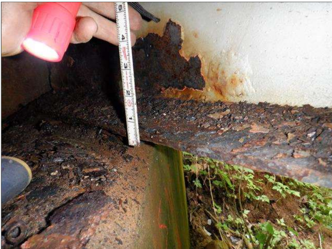
Span 3 Beam 9: [PAR] at far end, active corrosion with section loss; bottom flange [up to 38in x up to full width - avg rem 3/8in], lower web [up to 19in x up to 5in - avg rem 5/16in]
