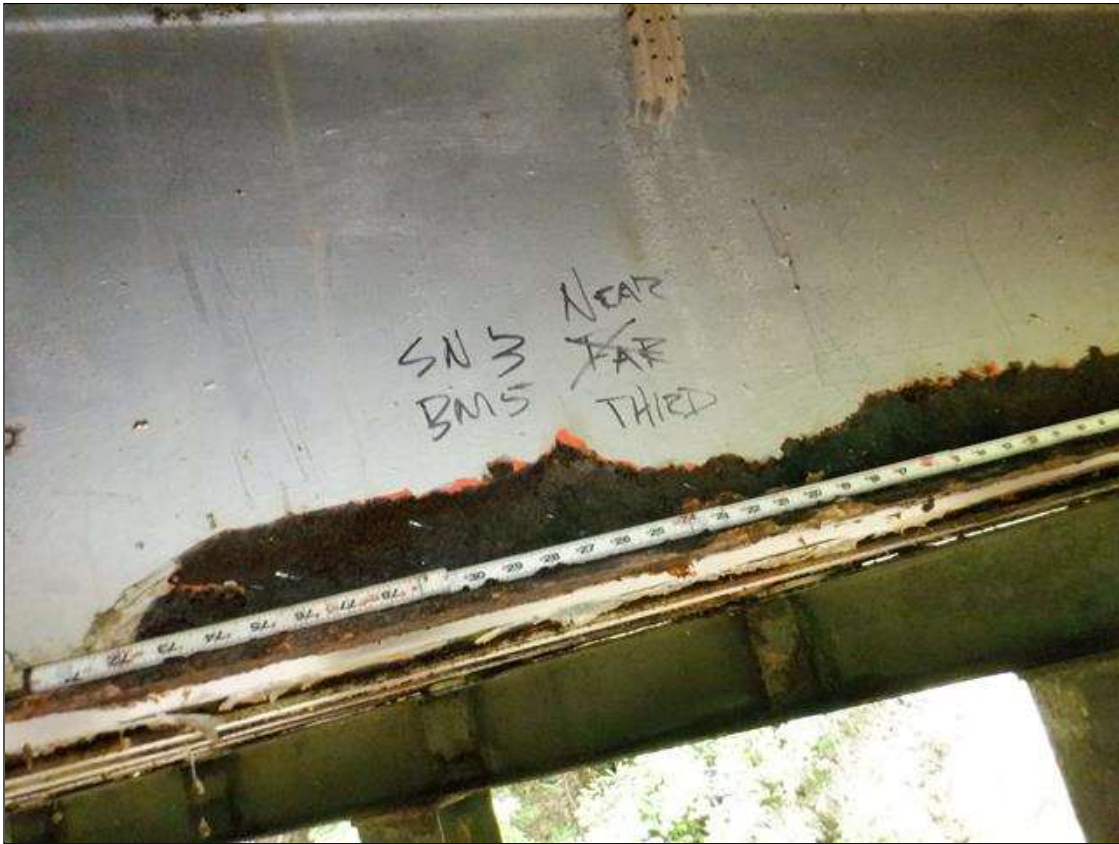
Span 3 Beam 5: [PAR] at near third, active corrosion with section loss; bottom flange [36in x up to full width - avg rem 3/8in], lower web [40in x up to 3in - avg rem 1/4in]
