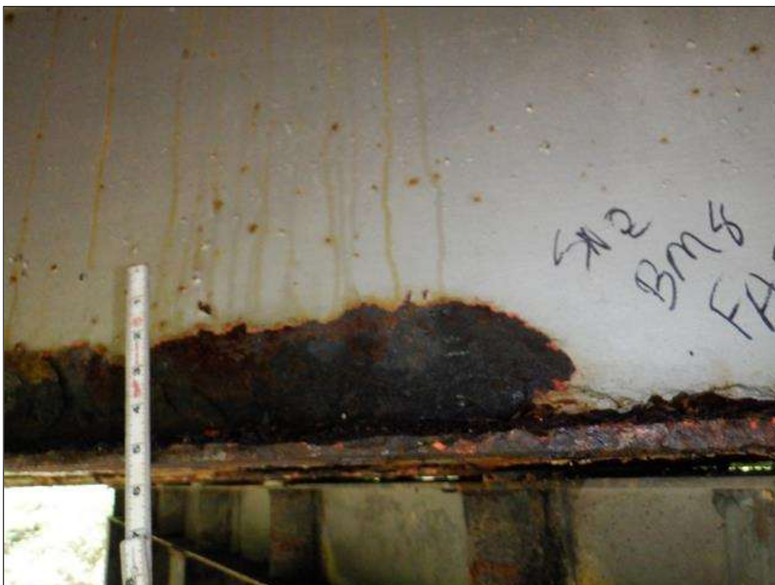
Span 2 Beam 8: [PAR] at 2ft from far end, active corrosion with section loss, South bottom flange [16in x 4in - avg rem 3/8in], lower web [28in x up to 2in - avg rem 1/4in]
