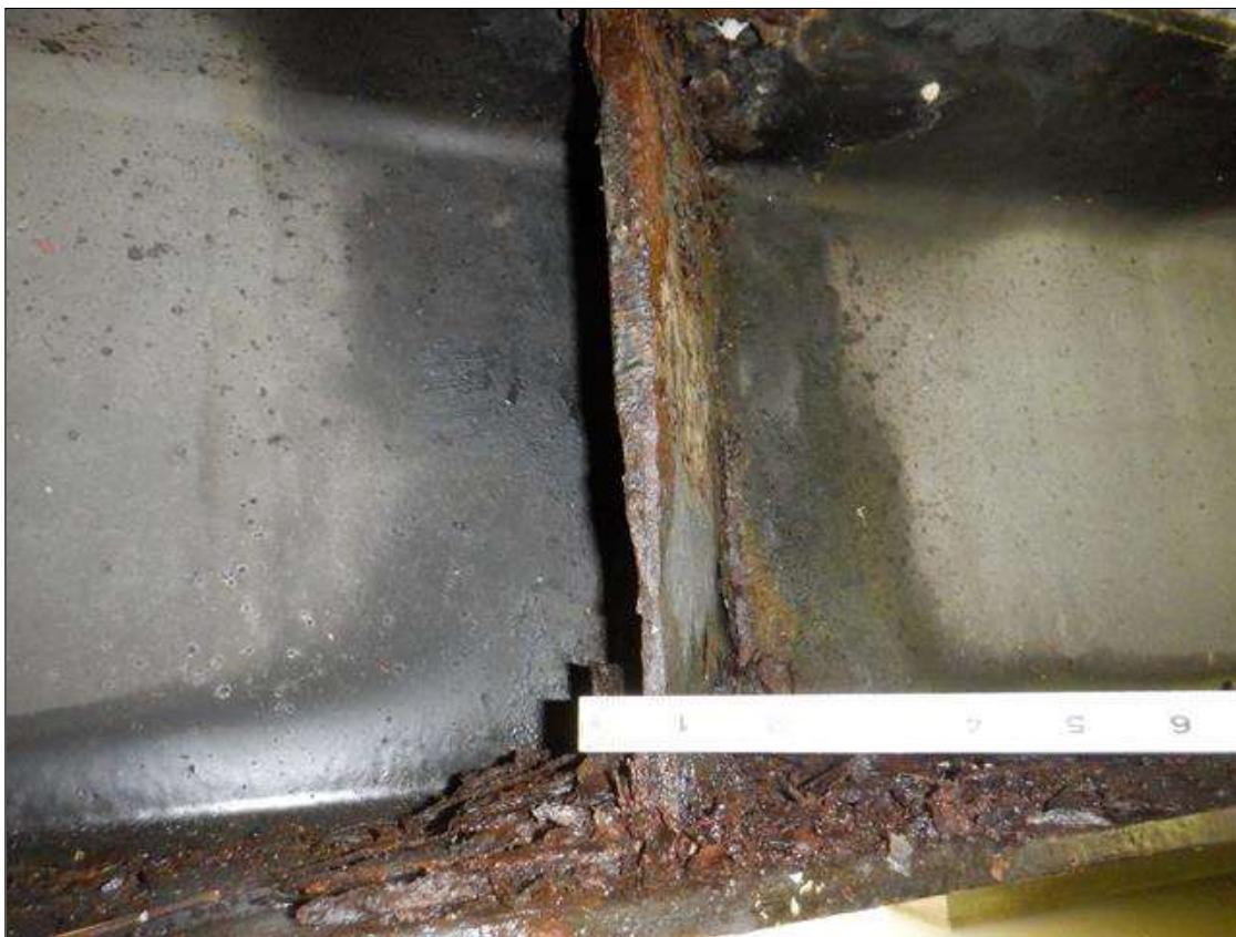
Bent 1 Cap 1: [PAR] along West face at stiffeners 2-6, 9, & 10, active corrosion with section loss [up to 6in x full width - avg rem 3/8in]; along East face at stiffeners 1-5, 9 & 10, active corrosion with section loss [8in x full width - avg rem 3/8in]
