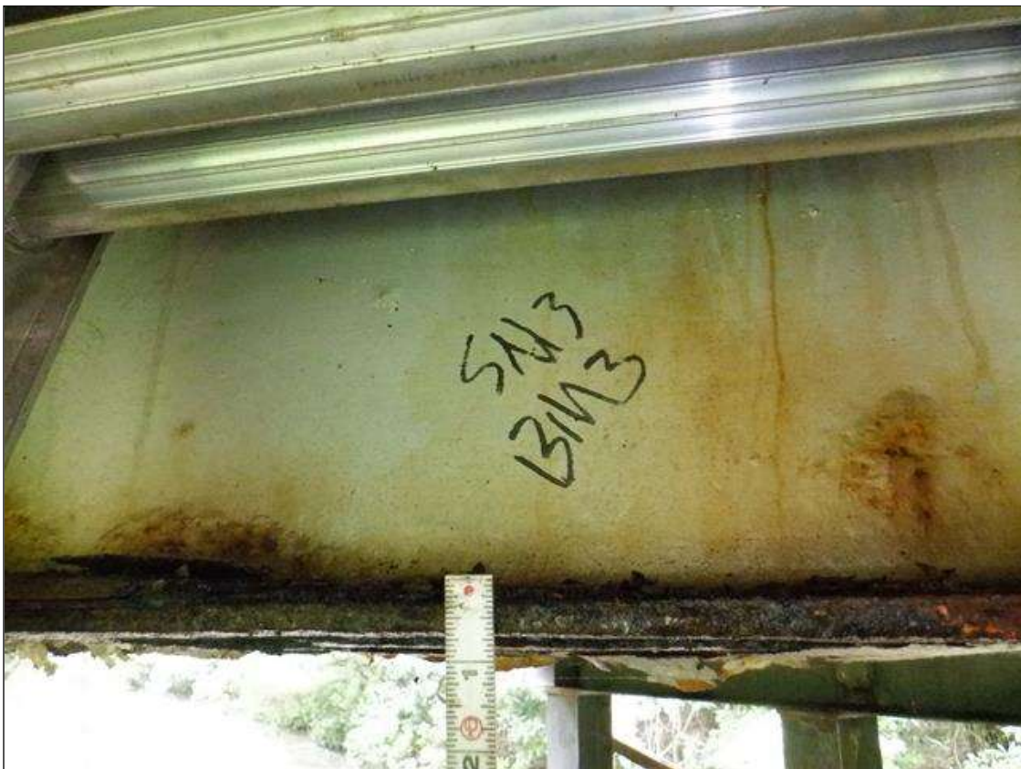
Span 3 Beam 3: [PAR] at midspan, active corrosion with section loss; bottom flange [up to 10ft x full width - avg rem 0.36in], lower web [up to 10ft x 4in - avg rem 5/16in]
