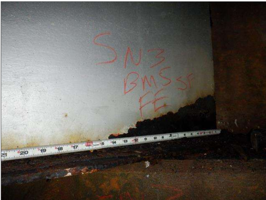
Span 3 Beam 5: [PAR] at far end, active corrosion with section loss, bottom flange [41in x full width - avg rem 3/8in], lower web [up to 24in x up to 4in - avg rem 5/16in]
