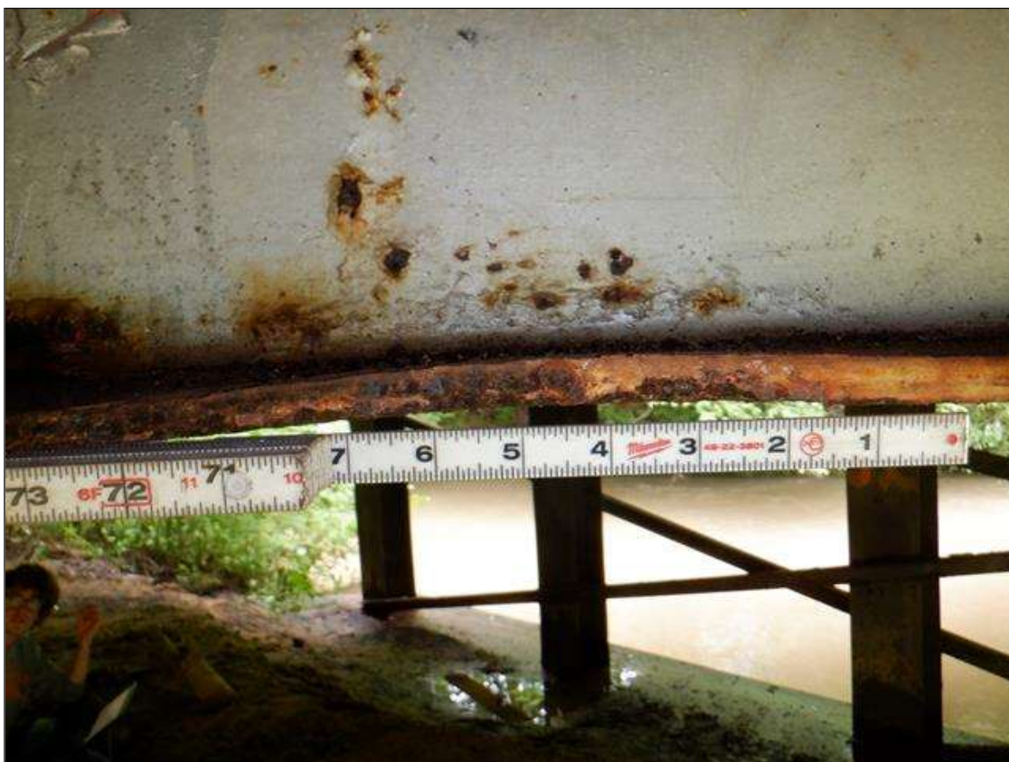
Span 1 Beam 9: South bottom flange at 2ft from interior diaphragm, distortion [6in x 1/4in]
