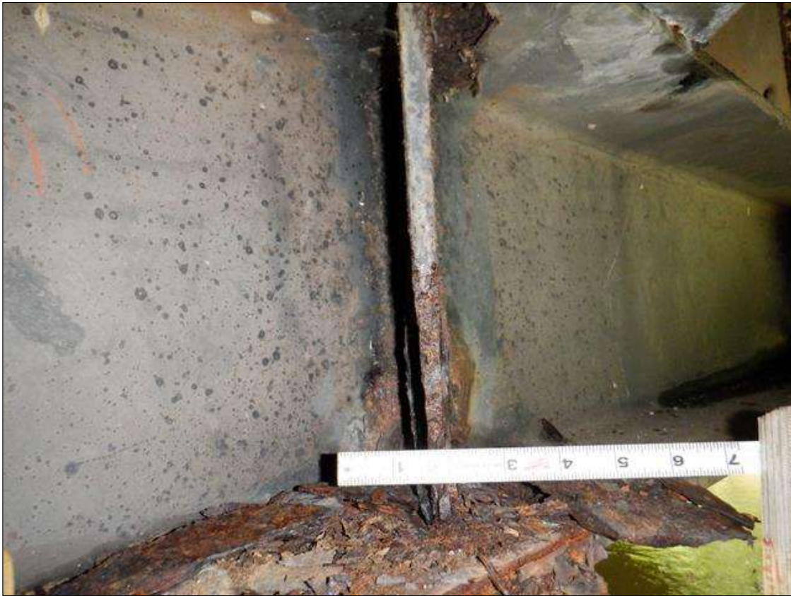
Bent 2 Cap 1: [PAR] along West face at stiffeners 2, 6, & 7, active corrosion with section loss [up to 6in x full width - avg rem 3/8in]; along East face at stiffeners 1, 2, & 7-9, active corrosion with section loss [8in x full width - avg rem 3/8in]
