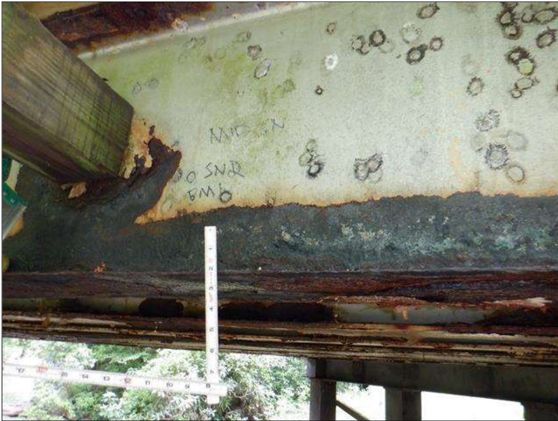
Span 2 Beam 1: [PAR] along length active corrosion with section loss; top and bottom flange [up to 15ft x full width - avg rem 3/8in], bottom flange at midspan [10ft x full width - avg rem 1/4in, with edges down to 1/8in], lower web along length [up to 15ft x up to 9in - avg rem 1/4in], lower web at midspan [10ft x 4in - avg rem 3/16in], web at rail connections [up to 12in diameter - avg rem 1/4in]
