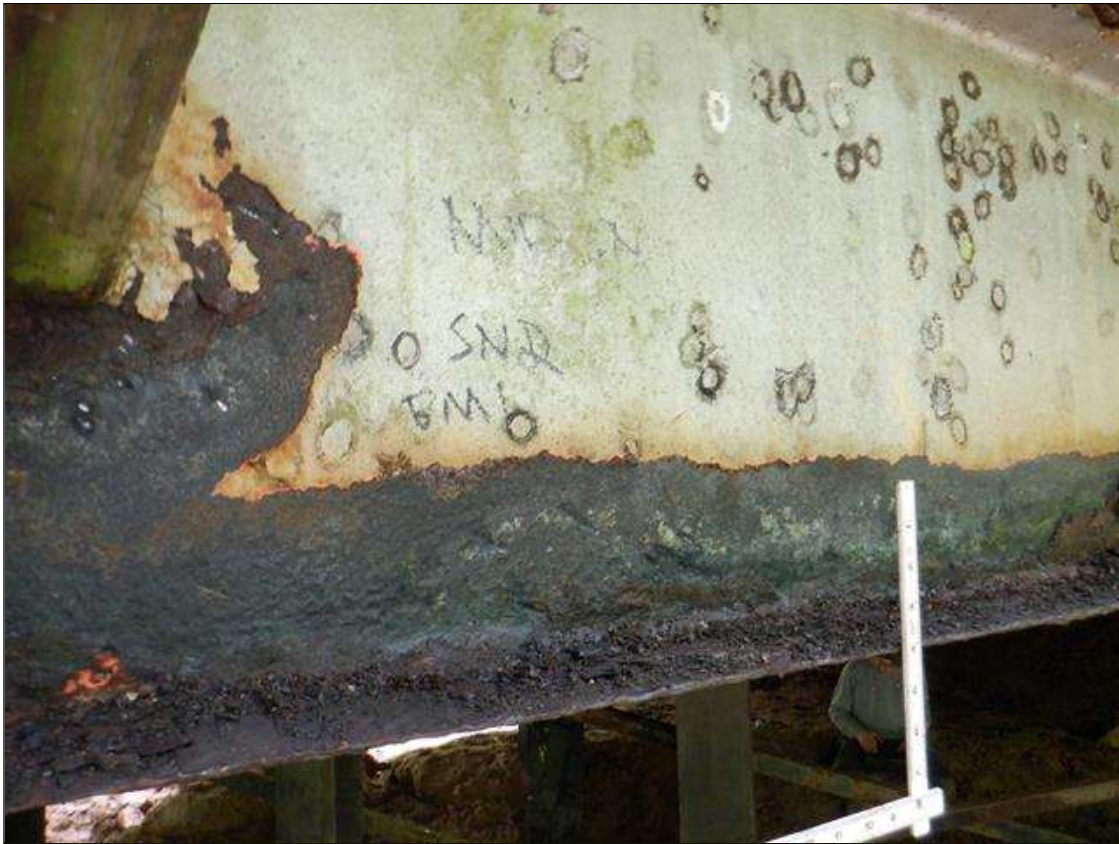
Span 2 Beam 1: [PAR] along length active corrosion with section loss; top and bottom flange [up to 15ft x full width - avg rem 3/8in], bottom flange at midspan [10ft x full width - avg rem 1/4in, with edges down to 1/8in], lower web along length [up to 15ft x up to 9in - avg rem 1/4in], lower web at midspan [10ft x 4in - avg rem 3/16in], web at rail connections [up to 12in diameter - avg rem 1/4in]
