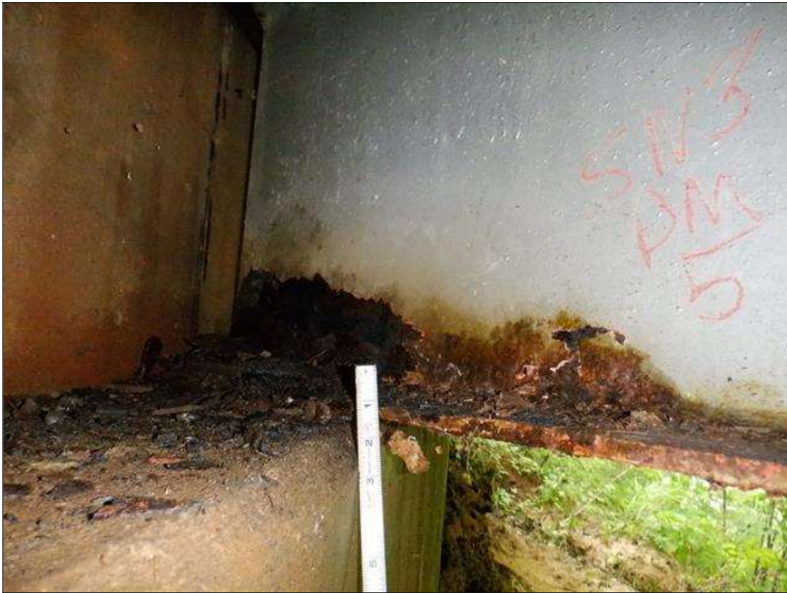
Span 3 Beam 5: [PAR] at far end, active corrosion with section loss, bottom flange [41in x full width - avg rem 3/8in], lower web [up to 24in x up to 4in - avg rem 5/16in]
