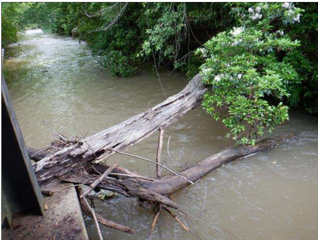
Drift: at bent 2 and West streambank, drift accumulation [up to 20in diameter]
