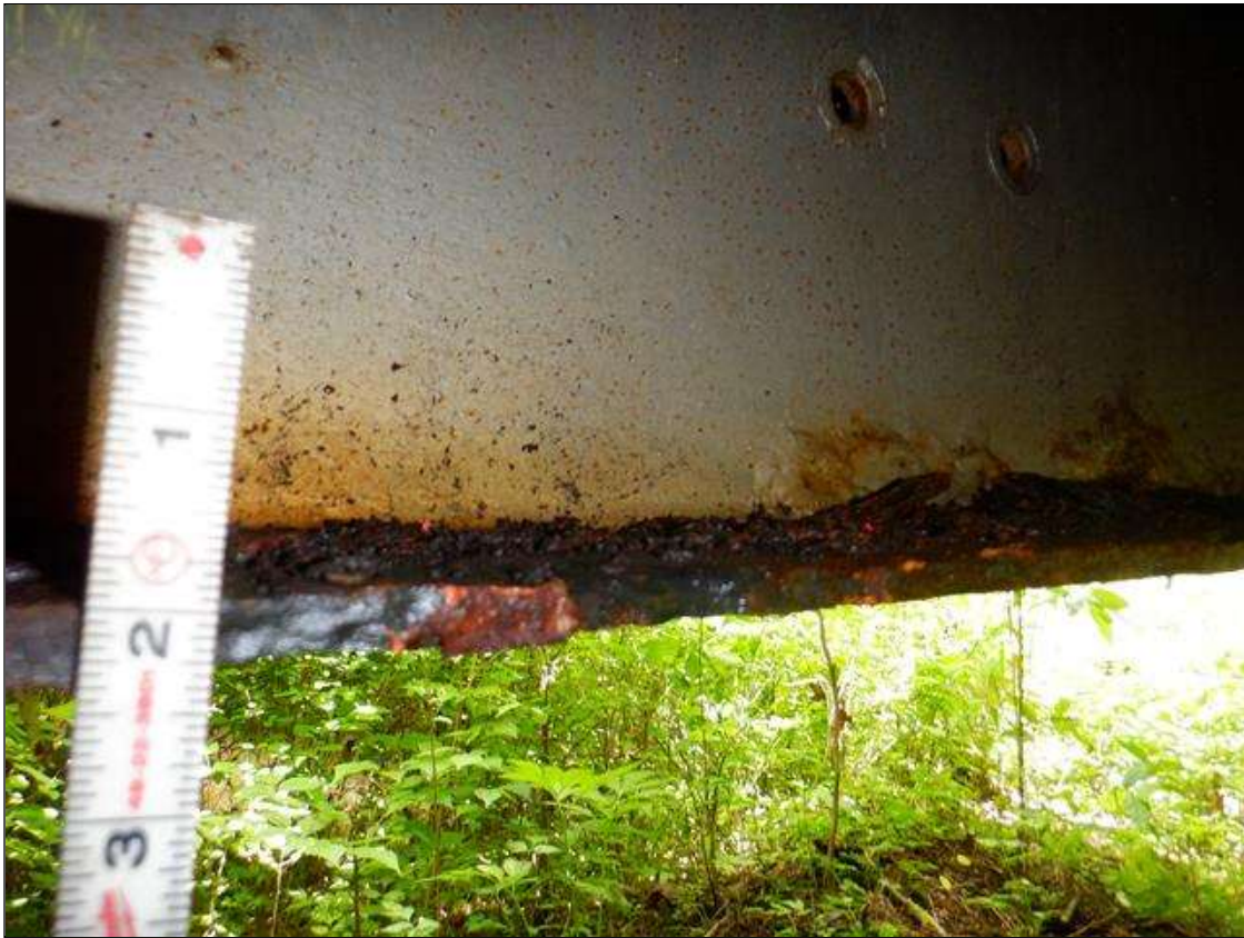
Span 1 Beam 2: [PAR] along length, active corrosion with section loss; top and bottom flange [full length x up to full width - avg rem 0.35in], lower web [up to 3ft x up to 6in - avg rem 5/16in]
