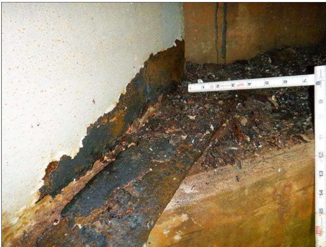
Span 1 Beam 4 Near Bearing: [PAR] North anchor bolt missing
