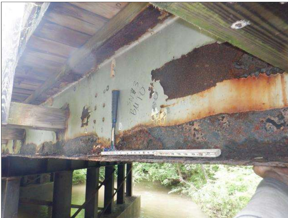
Span 3 Beam 10: [PAR] along length, active corrosion with section loss; top and bottom flange [full length x up to full width - avg rem 1/4in, with edges down to 1/16in], lower web [full length x up to 4in - avg rem 1/4in, with areas down to 3/16in], web at rail attachments [12in diameter - avg rem 1/4in]
