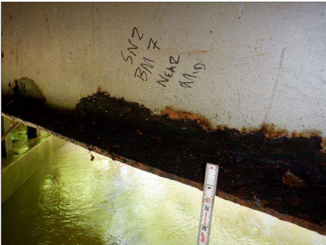
Span 2 Beam 7: [PAR] near midspan, active corrosion with section loss; bottom flange [up to 6ft x full width - avg rem 0.31in], lower web [up to 5ft x 2in - avg rem 5/16in]
