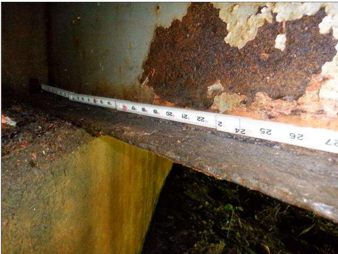
Span 1 Beam 8: [PAR] at near end, active corrosion with section loss; bottom flange [22in x full width - avg rem 1/4in], lower web [28in x up to 2-1/2in - avg rem 1/4in]
