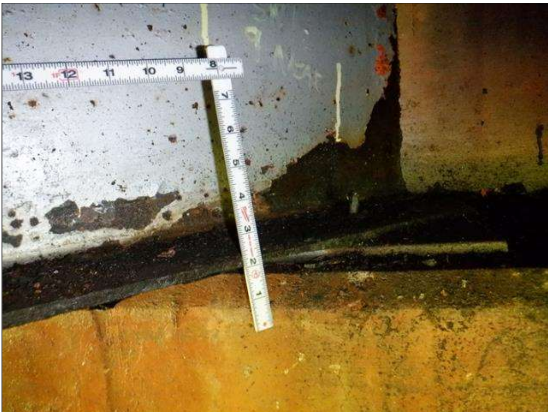
Span 1 Beam 9: [PAR] at near end, active corrosion with section loss; bottom flange [18in x full width - avg rem 0.35in], lower web [8in x up to 8in - avg rem 1/4in]
