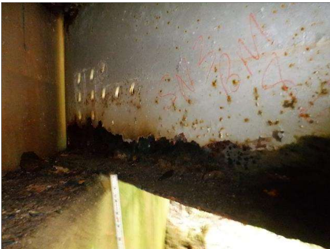
Span 3 Beam 8: [PAR] at far end, active corrosion with section loss; bottom flange [up to 27in x full width - avg rem 3/8in], lower web [up to 7ft x up to 3in - avg rem 5/16in]
