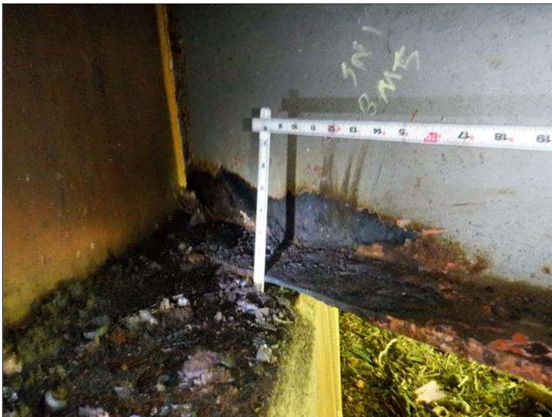
Span 1 Beam 5: [PAR] at near end, active corrosion with section loss; bottom flange [20in x full width - avg rem 3/8in], lower web [18in x 4in - avg rem 1/4in]
