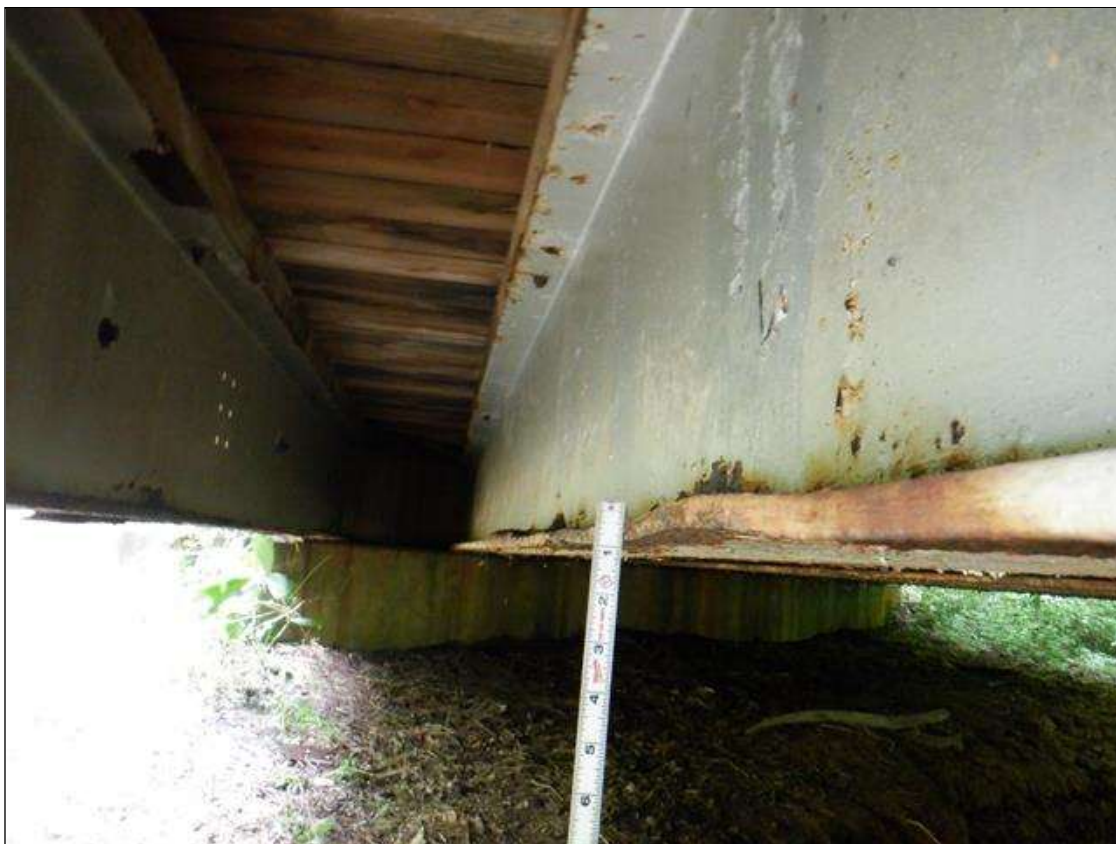
Span 1 Beam 9: South bottom flange at 2ft from interior diaphragm, distortion [6in x 1/4in]
