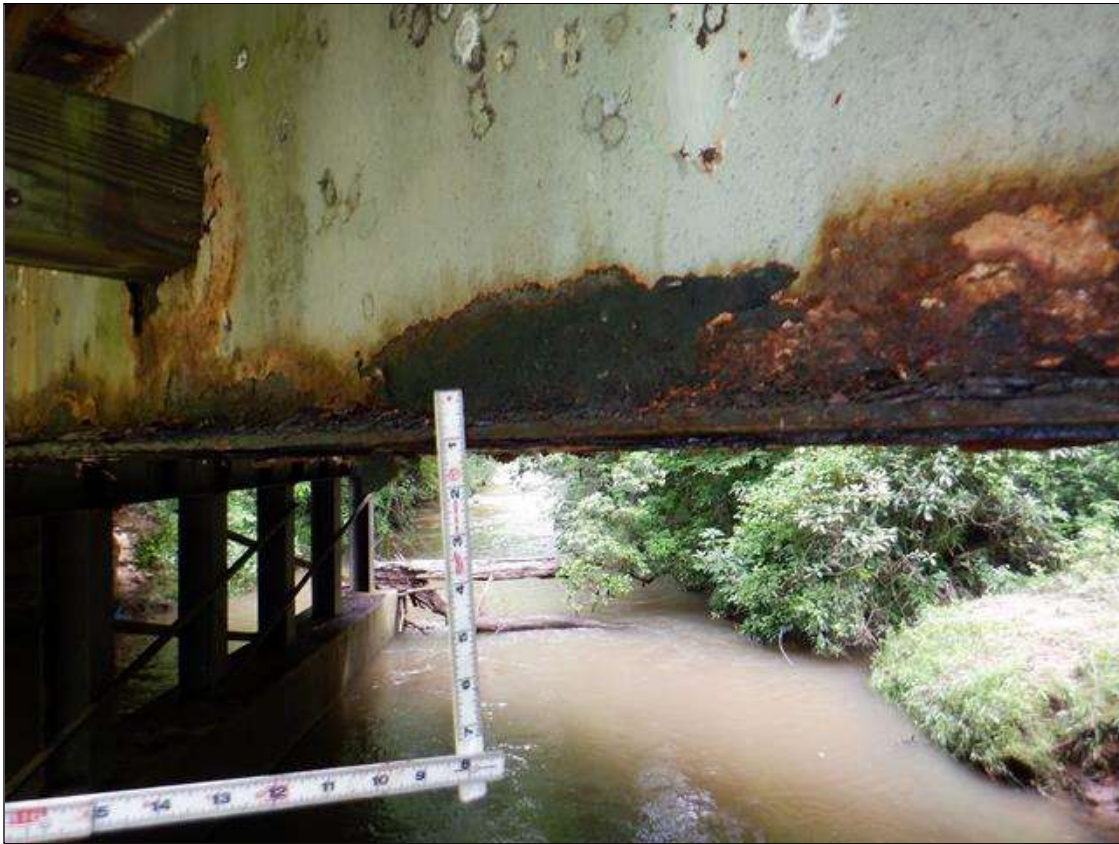
Span 2 Beam 1: [PAR] along length active corrosion with section loss; top and bottom flange [up to 15ft x full width - avg rem 3/8in], bottom flange at midspan [10ft x full width - avg rem 1/4in, with edges down to 1/8in], lower web along length [up to 15ft x up to 9in - avg rem 1/4in], lower web at midspan [10ft x 4in - avg rem 3/16in], web at rail connections [up to 12in diameter - avg rem 1/4in]
