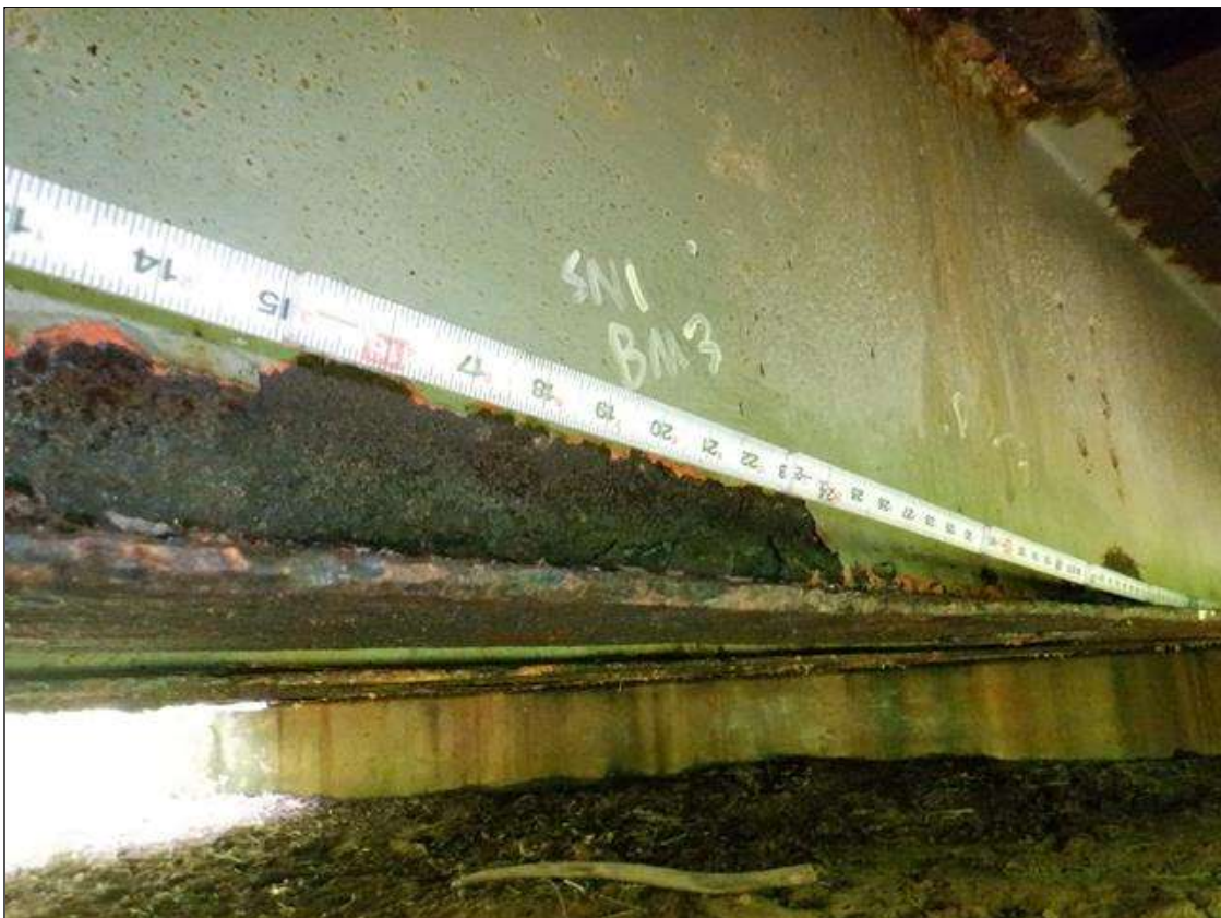
Span 1 Beam 3: [PAR] near midspan and at far third ,two [2] areas of active corrosion with section loss; bottom flange [up to 48in x full width - avg rem 3/8in], lower web [32in x 2-1/2in - avg rem 9/32in]
