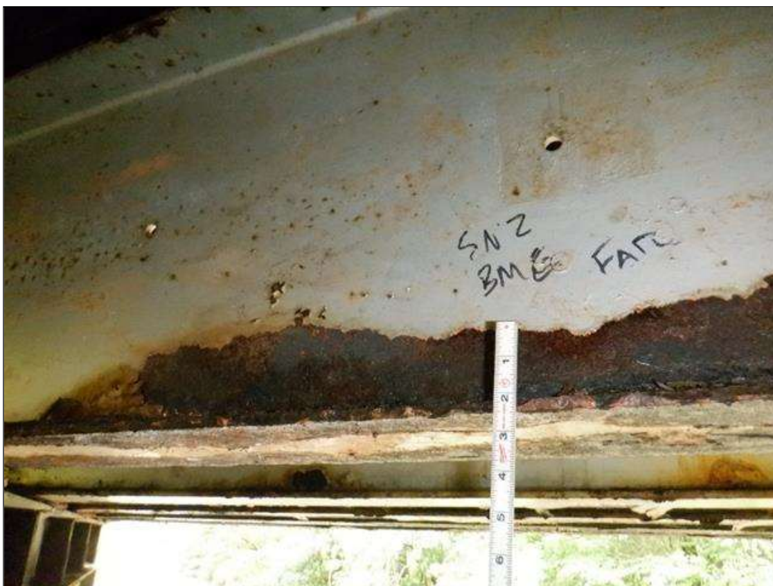
Span 2 Beam 6: [PAR] at far end, active corrosion with section loss; bottom flange [up to 8ft x full width - avg rem 3/8in], lower web [12ft x up to 2in - avg rem 1/4in]
