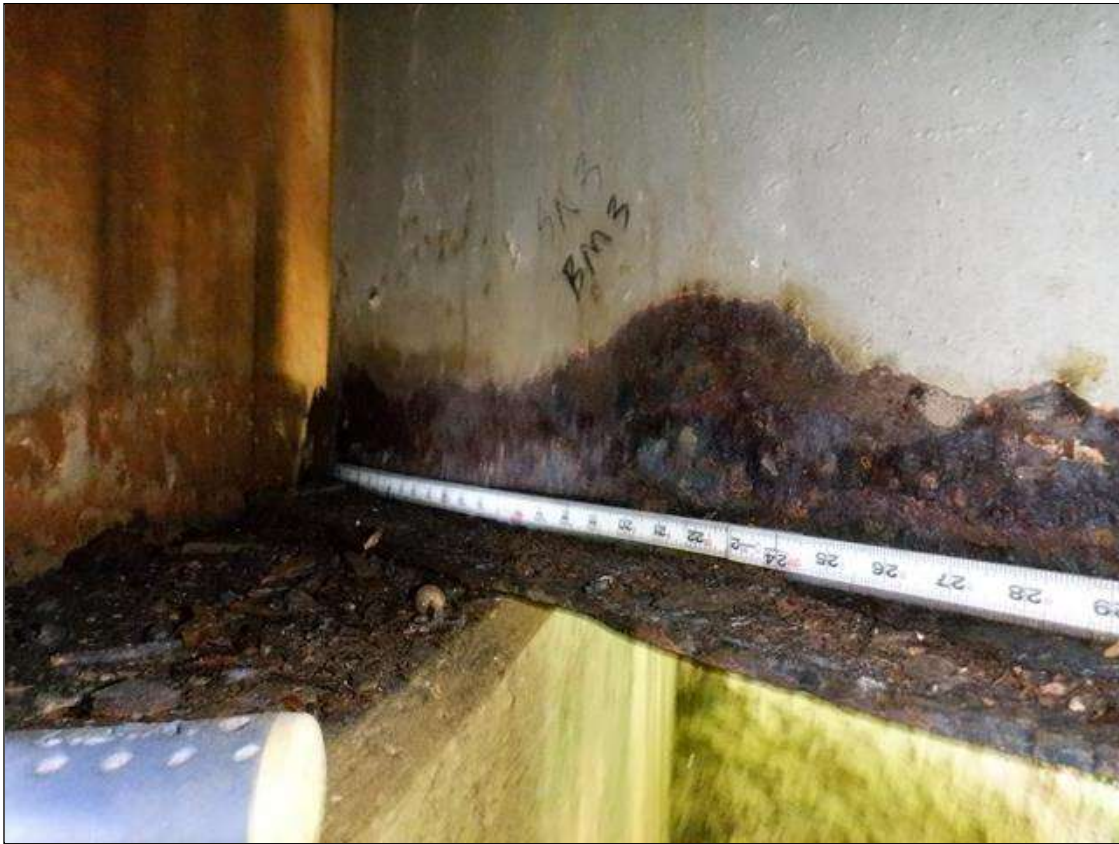
Span 3 Beam 3: [PAR] at far end, active corrosion with section loss; bottom flange [23in x up to full width - avg rem 3/8in], lower web [up to 32in x up to 5in - avg rem 5/16in]
