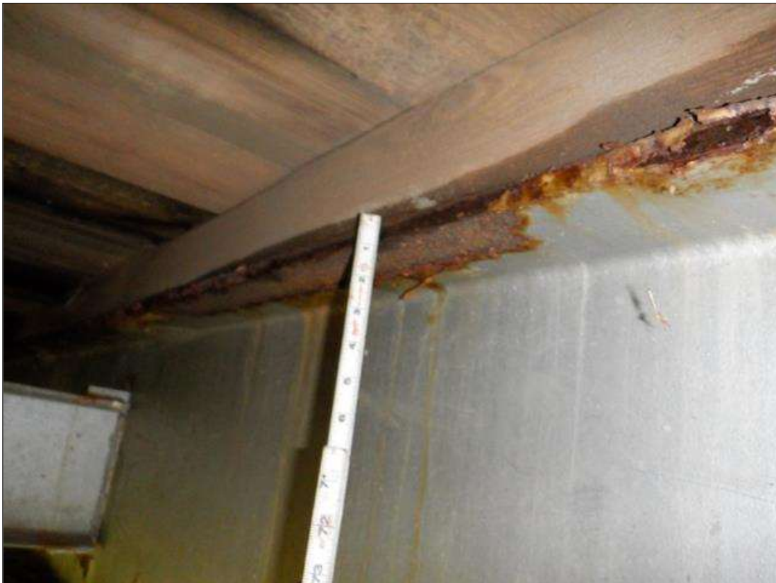
Span 3 Beam 4: [PAR] near midspan, active corrosion with section loss; top flange [up to 30in x up to full width - avg rem 5/16in], bottom flange [62in x up to full width - avg rem 7/16in]
