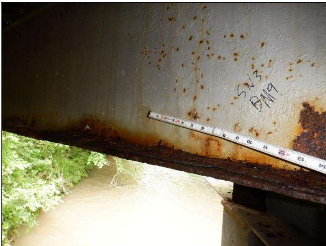
Span 3 Beam 9: [PAR] at near end, active corrosion with section loss; North bottom flange [41in x 4in - avg rem 3/8in]
