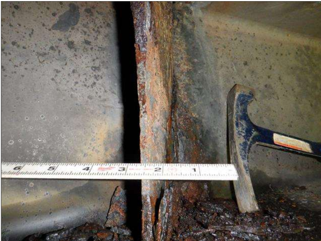
Bent 2 Cap 1: [PAR] along West face at stiffeners 2, 6, & 7, active corrosion with section loss [up to 6in x full width - avg rem 3/8in]; along East face at stiffeners 1, 2, & 7-9, active corrosion with section loss [8in x full width - avg rem 3/8in]
