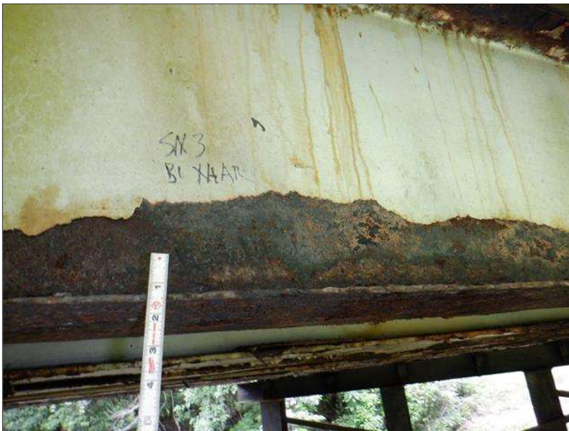
Span 3 Beam 1: [PAR] along length, active corrosion with section loss; top and bottom flange [full length x up to full width - avg rem 0.34in, edge down to 1/8in], lower and areas of upper web [16ft x up to 5in - avg rem 1/4in] , web at rail attachments [up to 12in diameter - avg rem 5/16in]
