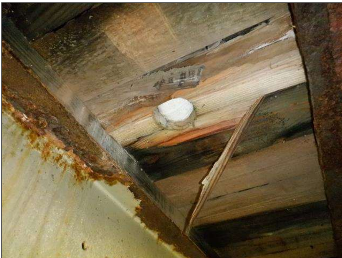
throughout underside of deck, multiple core holes [6in diameter]
