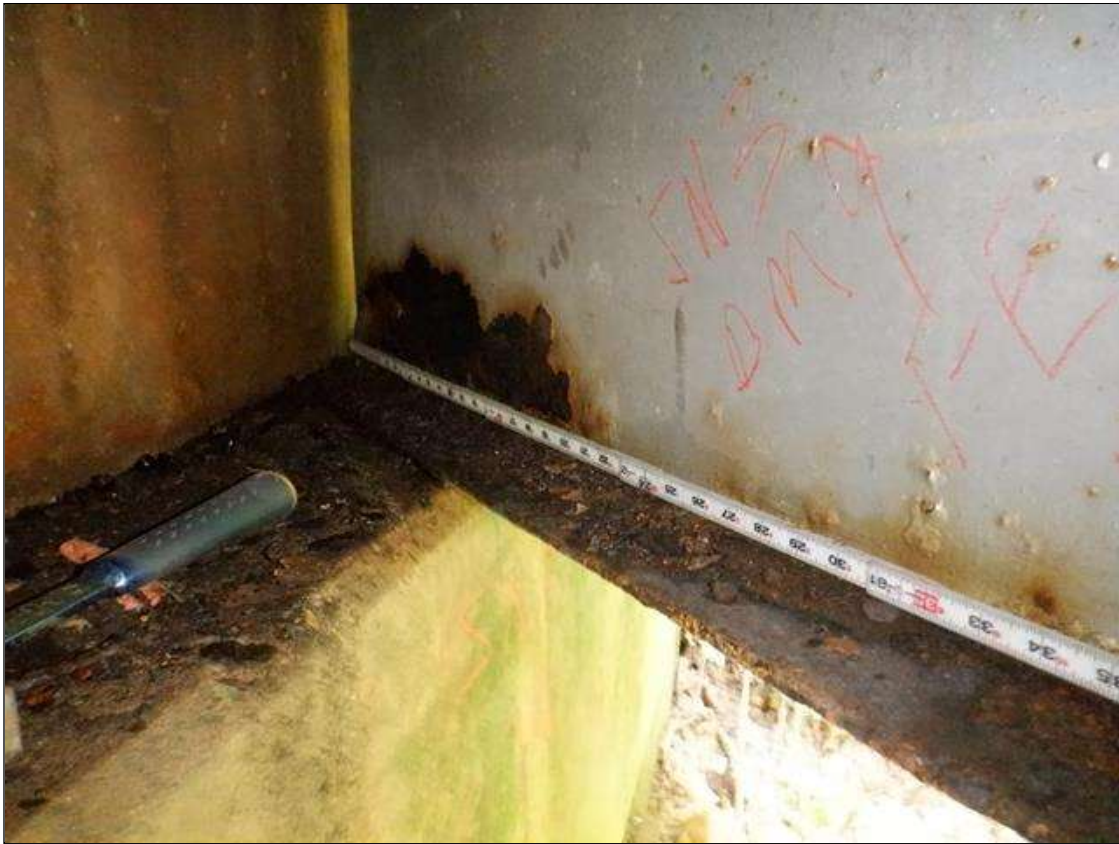
Span 3 Beam 9: [PAR] at far end, active corrosion with section loss; bottom flange [up to 38in x up to full width - avg rem 3/8in], lower web [up to 19in x up to 5in - avg rem 5/16in]
