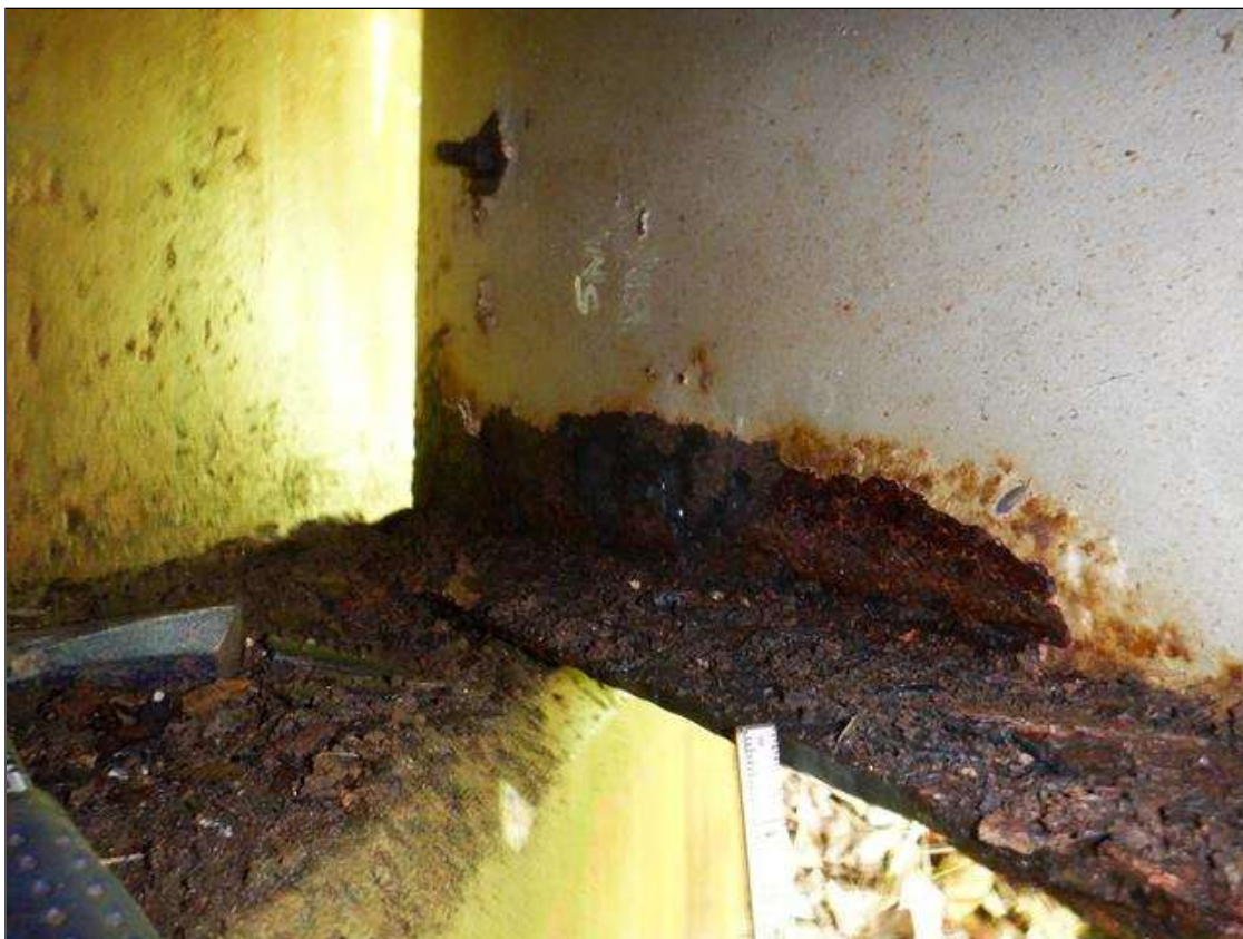
Span 1 Beam 1: [PAR] along length, active corrosion with section loss; top and bottom flange [full length x up to full width - avg rem 1/4in], lower web [full length x up to 3in - avg rem 5/16in]
