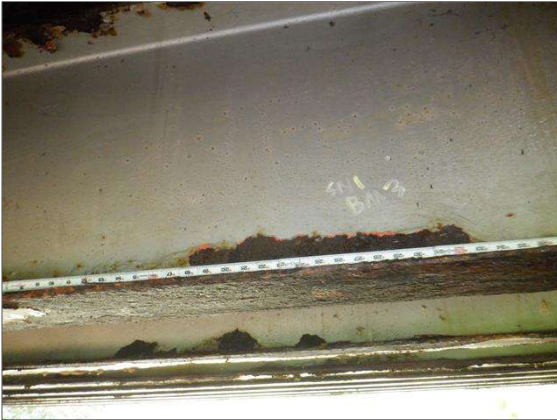
Span 1 Beam 3: [PAR] near midspan and at far third ,two [2] areas of active corrosion with section loss; bottom flange [up to 48in x full width - avg rem 3/8in], lower web [32in x 2-1/2in - avg rem 9/32in]
