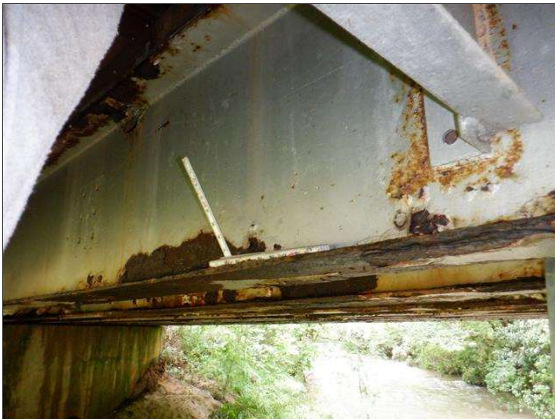
Span 3 Beam 2: [PAR] near midspan, active corrosion with section loss, bottom flange [10ft x full width - avg rem 0.35in], lower web [10ft x 4in - avg rem 5/16in]
