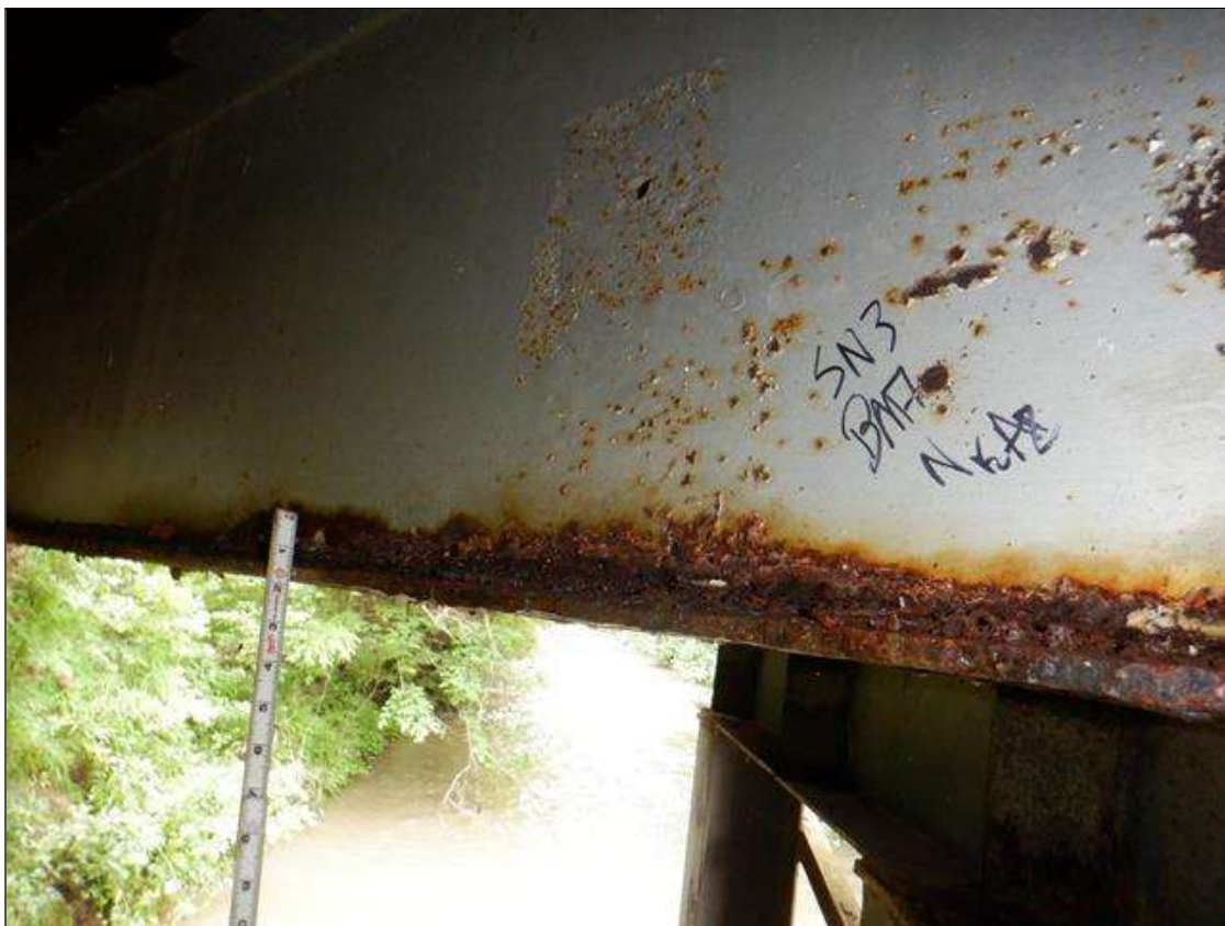
Span 3 Beam 7: [PAR] at 18in from near end, active corrosion with section loss; bottom flange [32in x up to full width - avg rem 3/8in]
