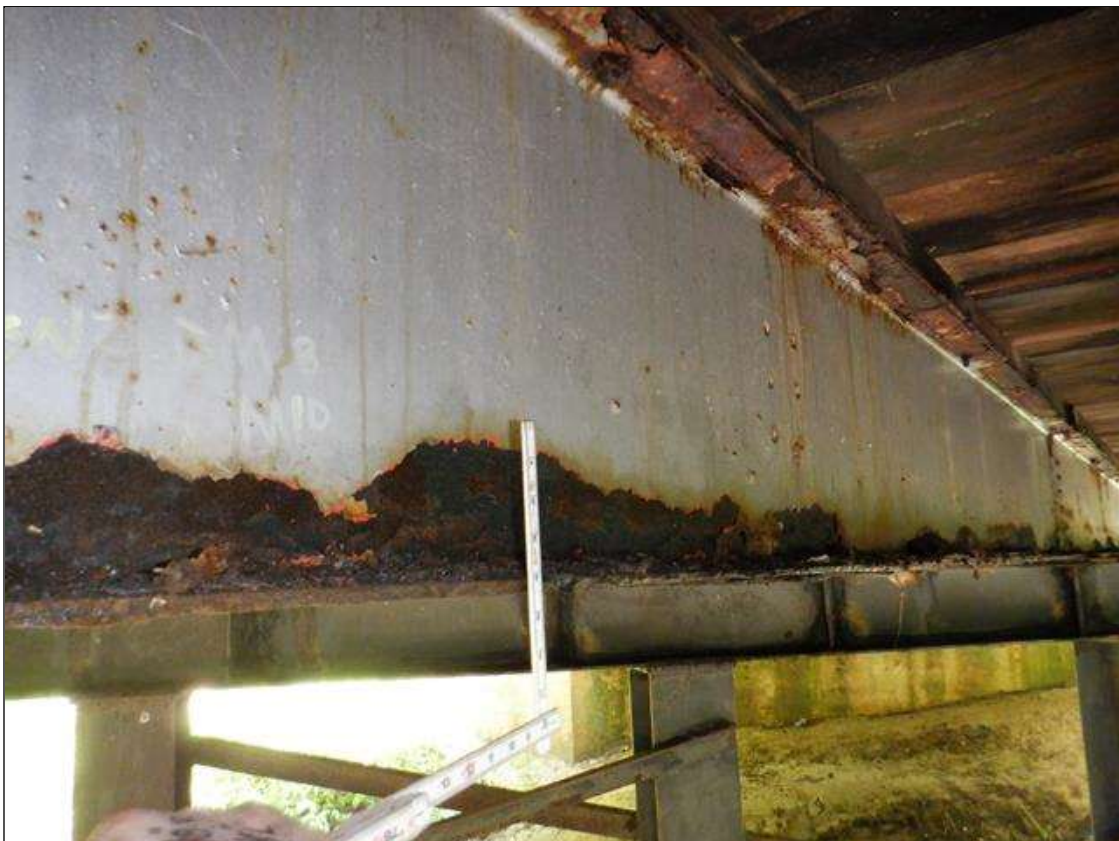
Span 2 Beam 8: [PAR] near midspan, active corrosion with section loss; top and bottom flange [63in x full width - avg rem 3/8in], lower web along length [up to 59in x up to 4in - avg rem 1/4in]
