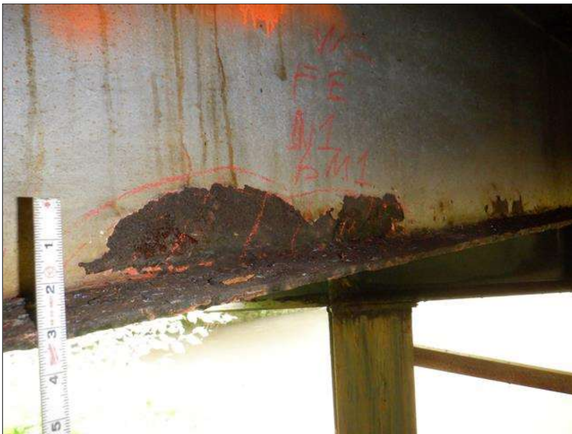
Span 1 Beam 1: [PAR] along length, active corrosion with section loss; top and bottom flange [full length x up to full width - avg rem 1/4in], lower web [full length x up to 3in - avg rem 5/16in]
