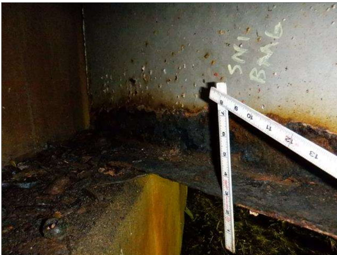
Span 1 Beam 6: [PAR] at near end, active corrosion with section loss, South bottom flange [up to 36in x up to 4in - avg rem 3/8in], lower web [30in x up to 3in - avg rem 1/4in]
