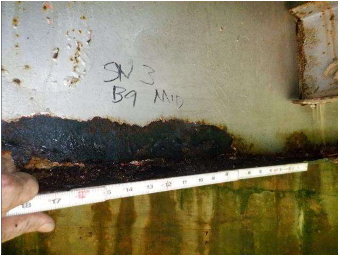
Span 3 Beam 9: [PAR] near midspan, active corrosion with section loss; bottom flange [24in x full width - avg rem 3/8in], lower web [20in x 2in - avg rem 1/4in]
