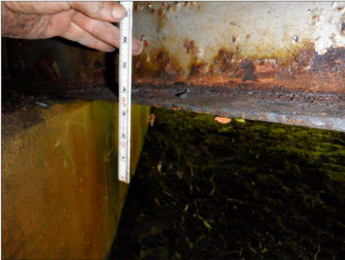
Span 1 Beam 7: [PAR] bottom flange at near end, active corrosion with section loss [up to 30in x up to full width - avg rem 3/8in, with areas down to 1/4in at edges]
