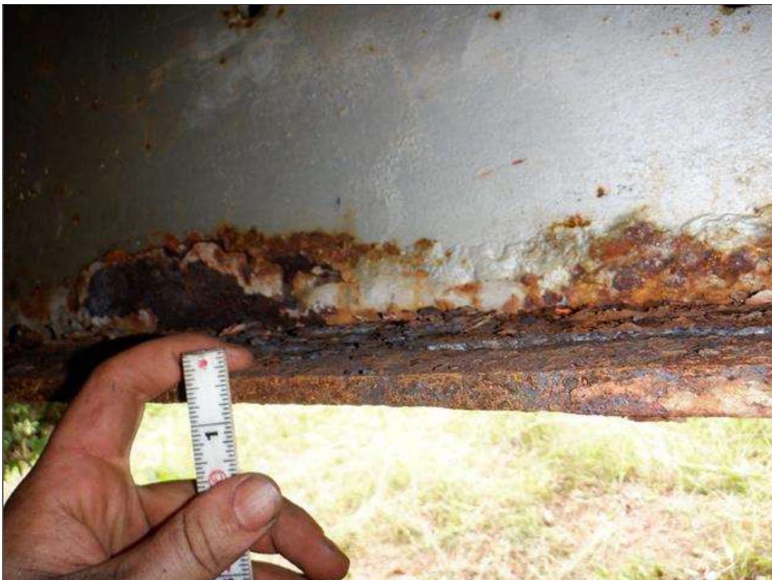
Span 1 Beam 8: 2ft from far end, active corrosion with section loss; top and bottom flange [9ft x up to full width - avg rem 7/16in], lower web [up to 3ft x up to 4in - avg rem 5/16in]
