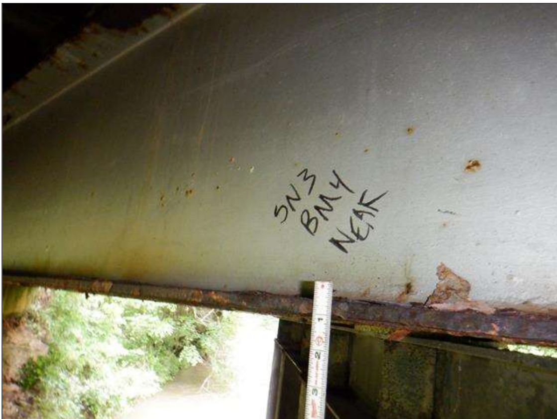
Span 3 Beam 4: [PAR] at near end, active corrosion with section loss; North bottom flange [4ft x 4in - avg rem 3/8in]
