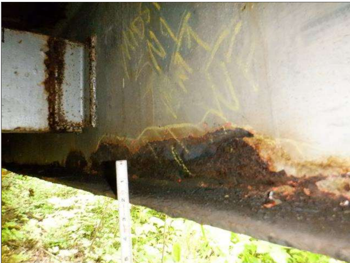
Span 1 Beam 1: [PAR] along length, active corrosion with section loss; top and bottom flange [full length x up to full width - avg rem 1/4in], lower web [full length x up to 3in - avg rem 5/16in]
