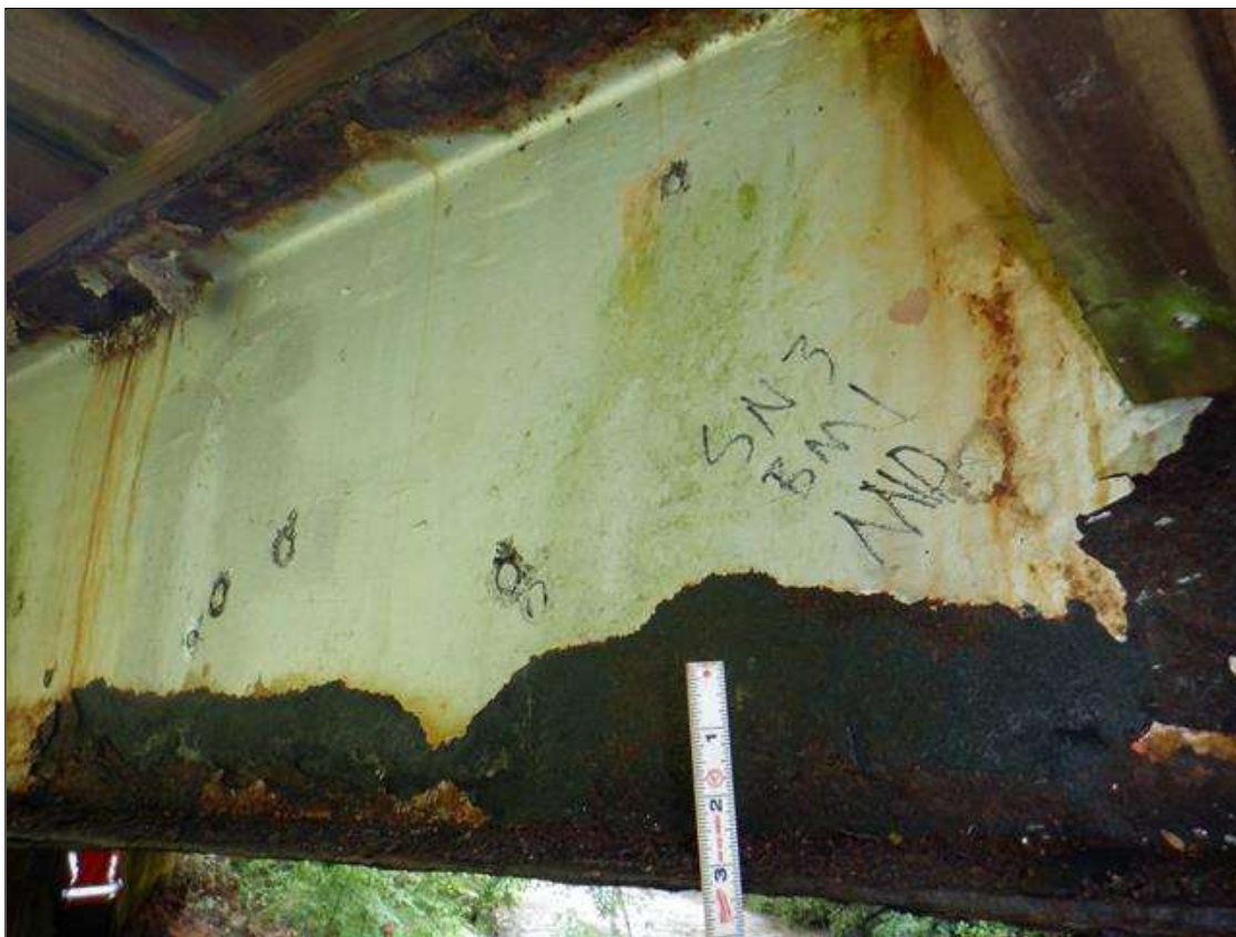
Span 3 Beam 1: [PAR] along length, active corrosion with section loss; top and bottom flange [full length x up to full width - avg rem 0.34in, edge down to 1/8in], lower and areas of upper web [16ft x up to 5in - avg rem 1/4in] , web at rail attachments [up to 12in diameter - avg rem 5/16in]
