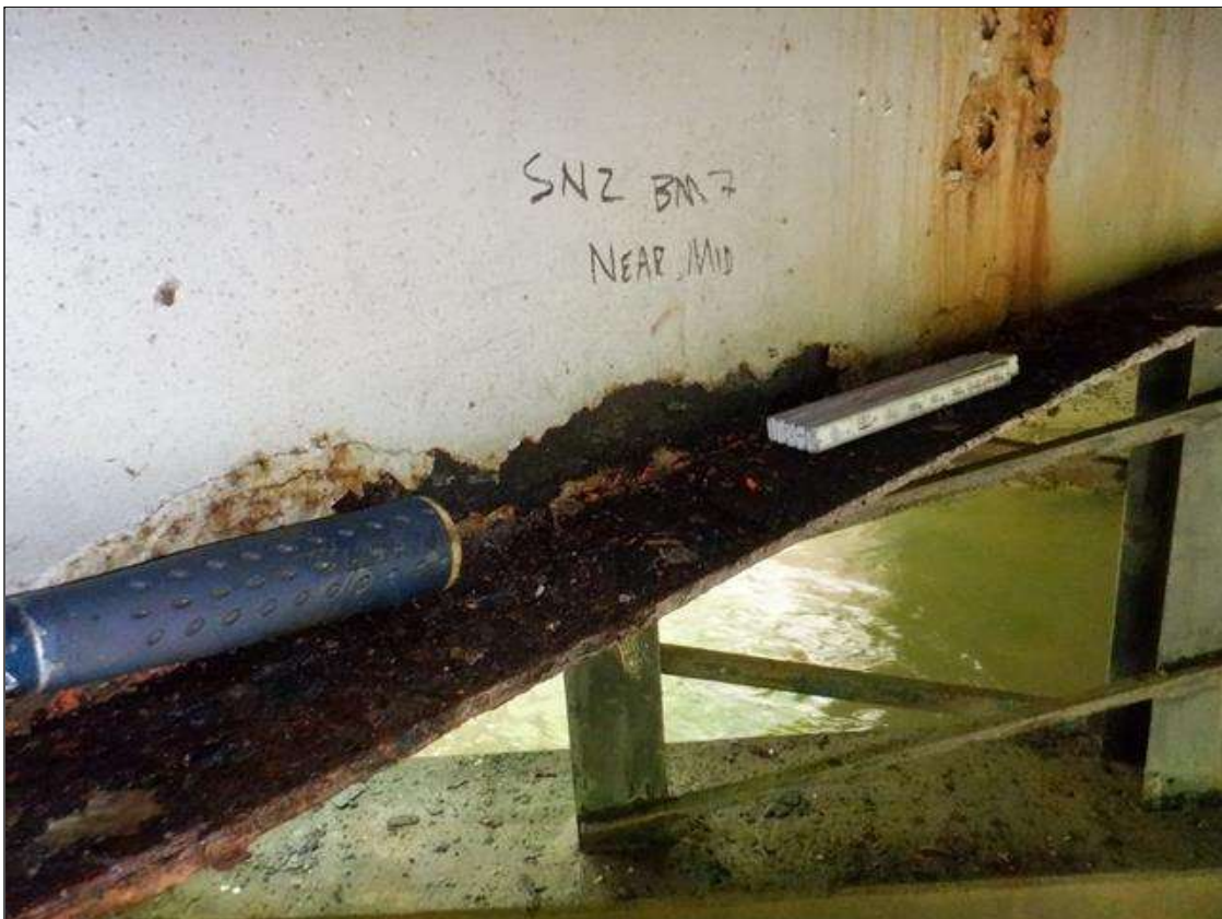
Span 2 Beam 7: [PAR] near midspan, active corrosion with section loss; bottom flange [up to 6ft x full width - avg rem 0.31in], lower web [up to 5ft x 2in - avg rem 5/16in]
