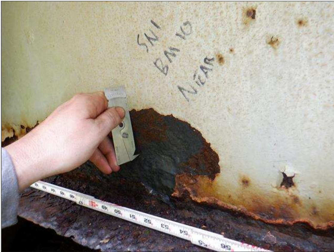
Span 1 Beam 10: [PAR] along length of beam, multiple areas of active corrosion with section loss; bottom flange [up to 68in x 6in - avg rem 1/4in], lower web & web at rail post connections [up to 10ft x 6in - avg rem 1/4in]
