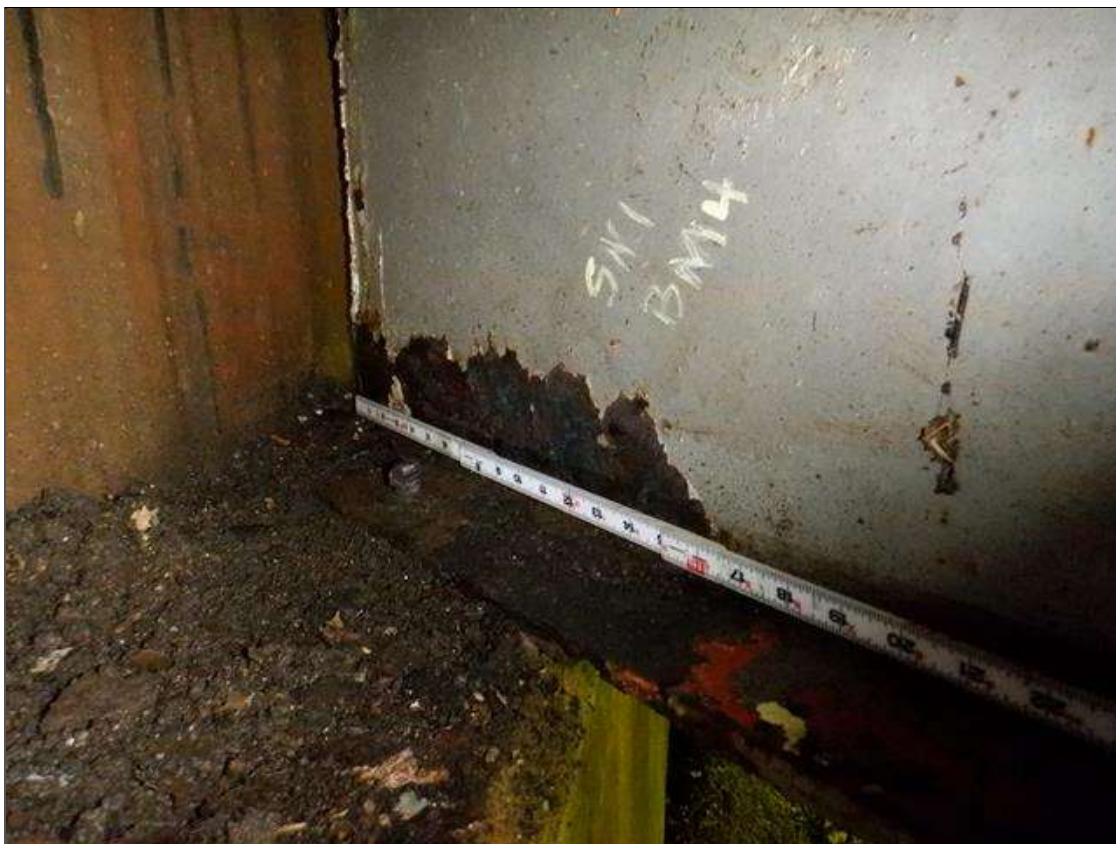
Span 1 Beam 4: [PAR] at near end, active corrosion with section loss; bottom flange [16in x full width - avg rem 1/2in], lower web [14in x 2in - avg rem 1/4in]
