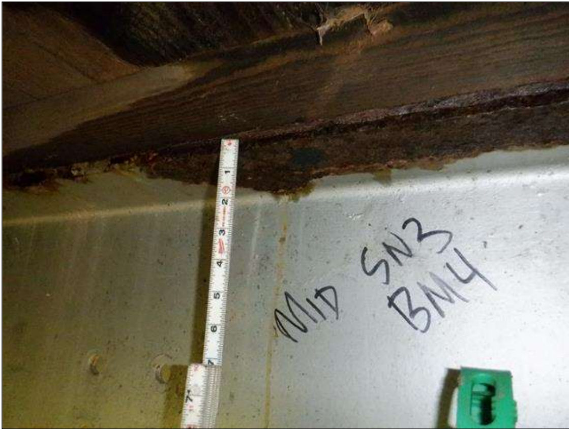
Span 3 Beam 4: [PAR] near midspan, active corrosion with section loss; top flange [up to 30in x up to full width - avg rem 5/16in], bottom flange [62in x up to full width - avg rem 7/16in]
