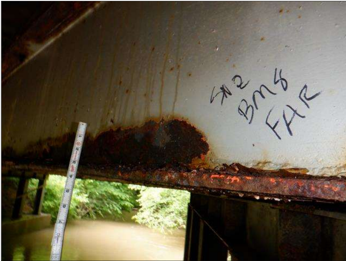
Span 2 Beam 8: [PAR] at 2ft from far end, active corrosion with section loss, South bottom flange [16in x 4in - avg rem 3/8in], lower web [28in x up to 2in - avg rem 1/4in]
