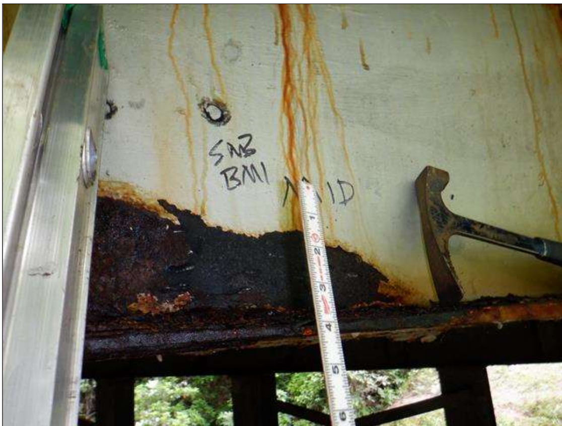
Span 3 Beam 1: [PAR] along length, active corrosion with section loss; top and bottom flange [full length x up to full width - avg rem 0.34in, edge down to 1/8in], lower and areas of upper web [16ft x up to 5in - avg rem 1/4in], web at rail attachments [up to 12in diameter - avg rem 5/16in]
