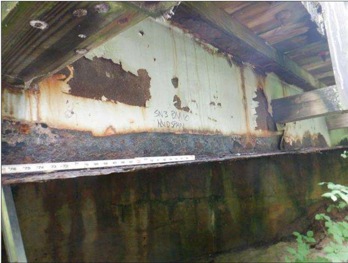
Span 3 Beam 10: [PAR] along length, active corrosion with section loss; top and bottom flange [full length x up to full width - avg rem 1/4in, with edges down to 1/16in], lower web [full length x up to 4in - avg rem 1/4in, with areas down to 3/16in], web at rail attachments [12in diameter - avg rem 1/4in]
