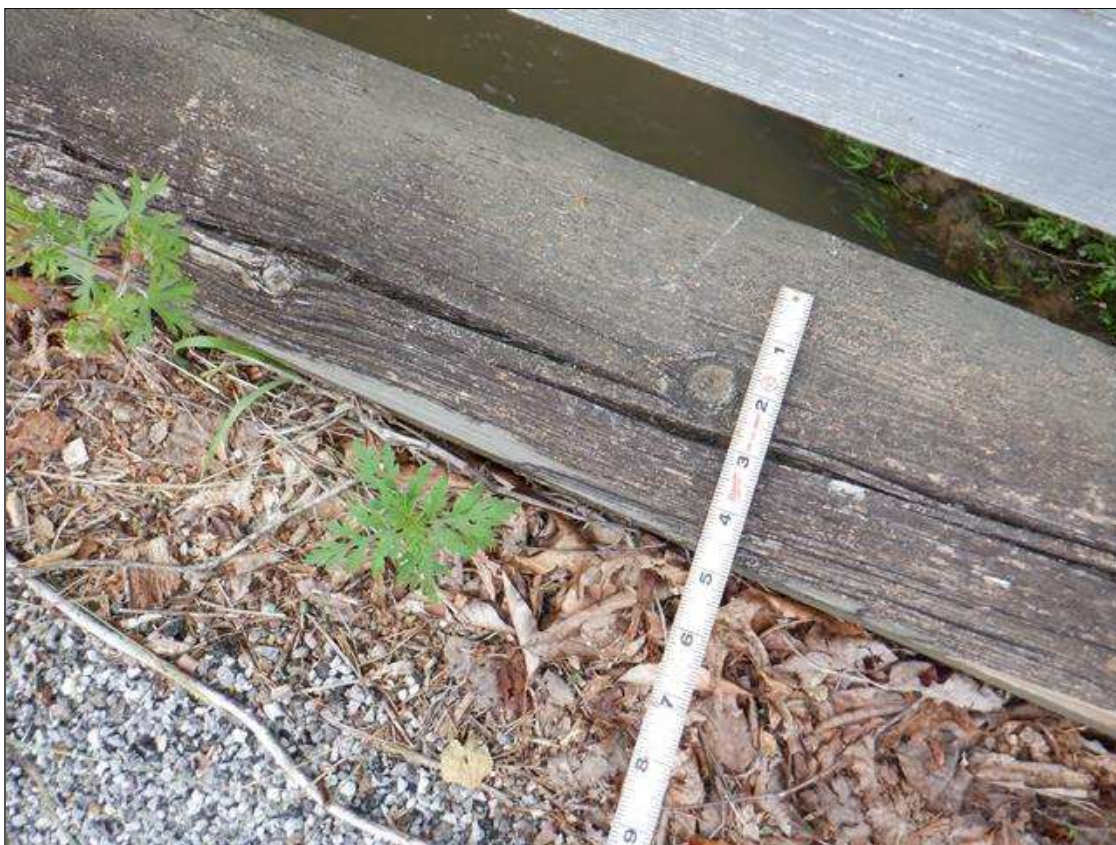
Span 3 Left Bridge Rail: top board and curb, checks (full length x up to 1/4in)
