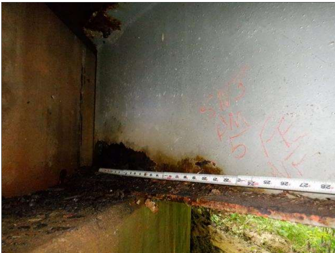
Span 3 Beam 5: [PAR] at far end, active corrosion with section loss, bottom flange [41in x full width - avg rem 3/8in], lower web [up to 24in x up to 4in - avg rem 5/16in]
