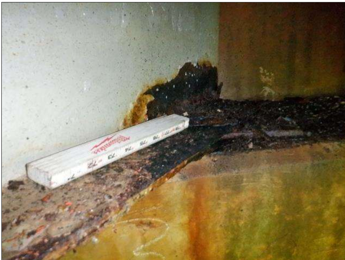
Span 1 Beam 3 Near Bearing: [PAR] North anchor bolt missing
