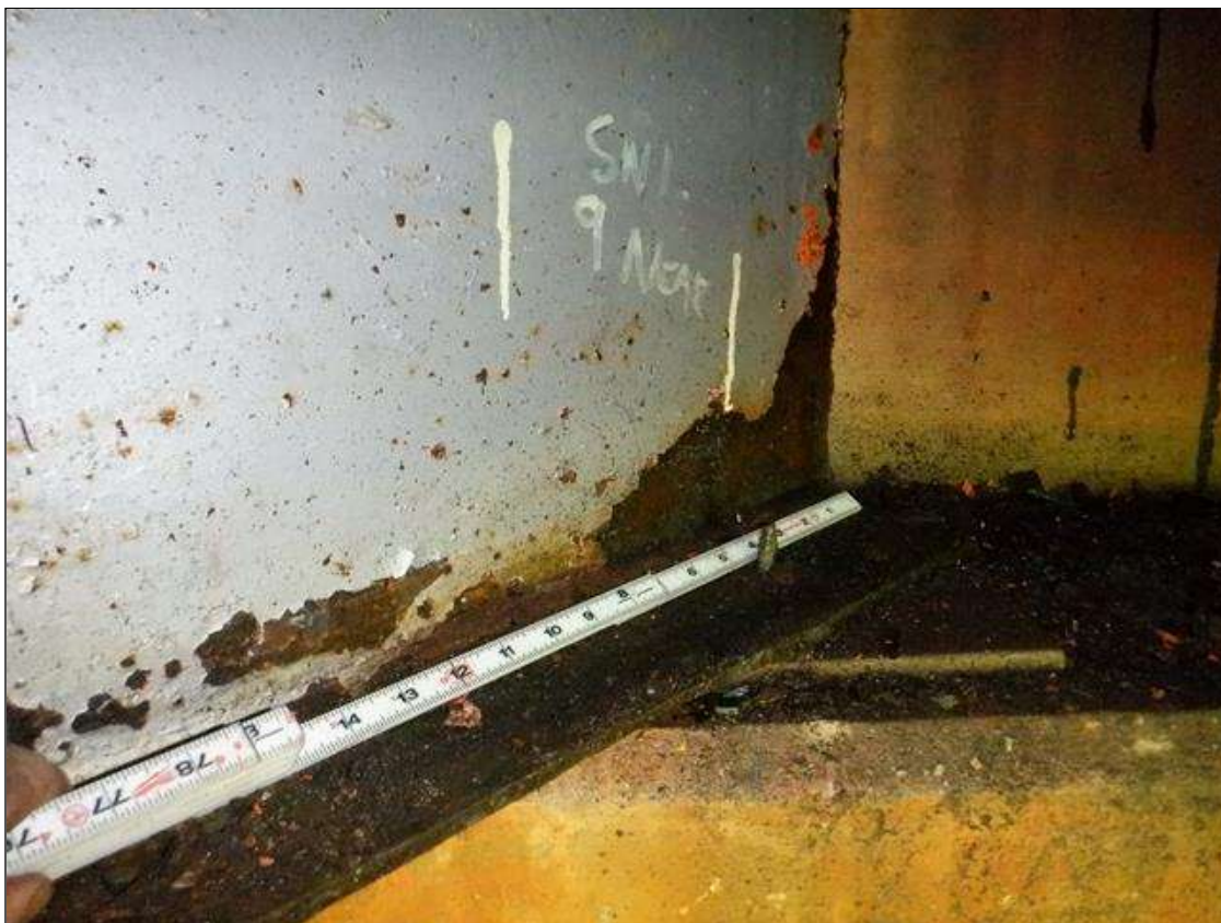
Span 1 Beam 9: [PAR] at near end, active corrosion with section loss; bottom flange [18in x full width - avg rem 0.35in], lower web [8in x up to 8in - avg rem 1/4in]
