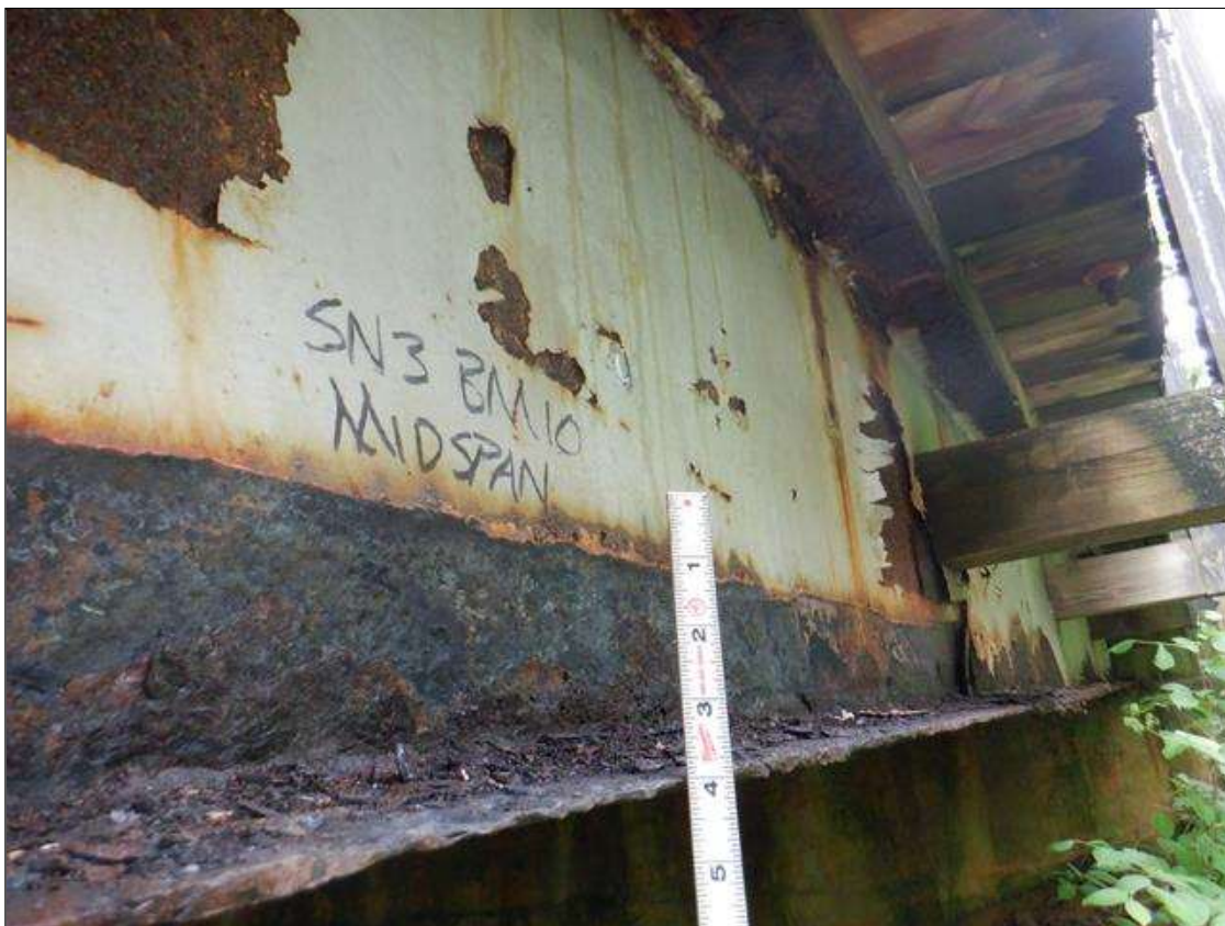
Span 3 Beam 10: [PAR] along length, active corrosion with section loss; top and bottom flange [full length x up to full width - avg rem 1/4in, with edges down to 1/16in], lower web [full length x up to 4in - avg rem 1/4in, with areas down to 3/16in], web at rail attachments [12in diameter - avg rem 1/4in]
