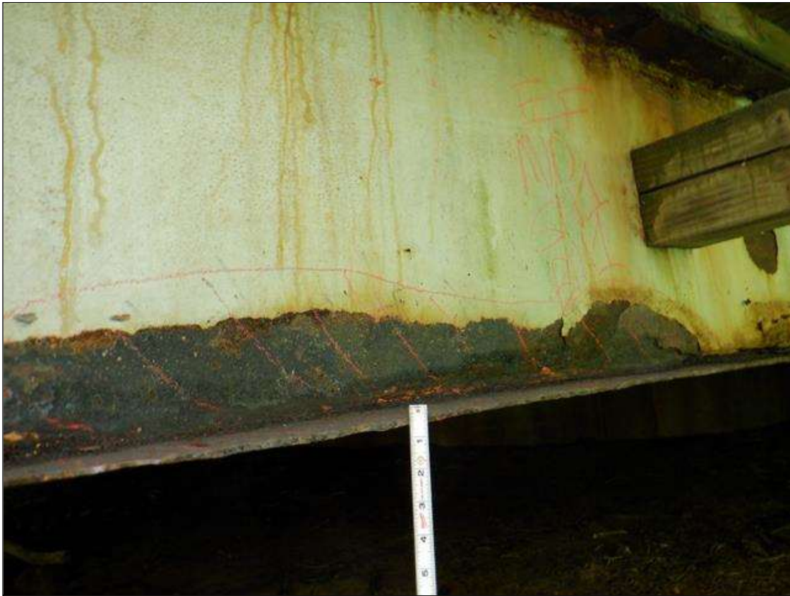
Span 1 Beam 1: [PAR] along length, active corrosion with section loss; top and bottom flange [full length x up to full width - avg rem 1/4in], lower web [full length x up to 3in - avg rem 5/16in]
