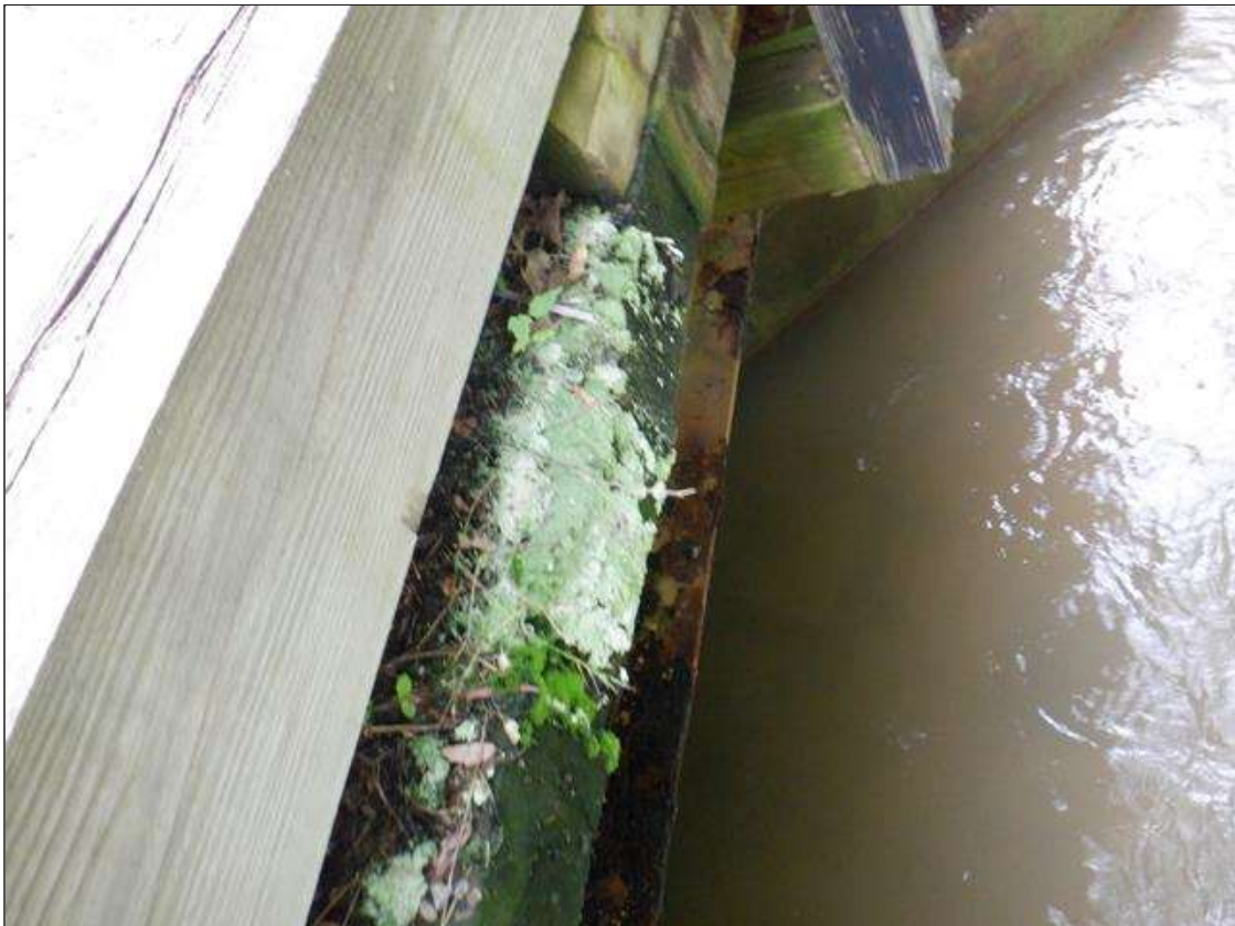
Span 3 Deck: throughout edge of deck at North and South ends, areas of decay/surface softness in end of deck boards [up to full width x full height x up to 1in deep probe] with vegetation/moss growth
