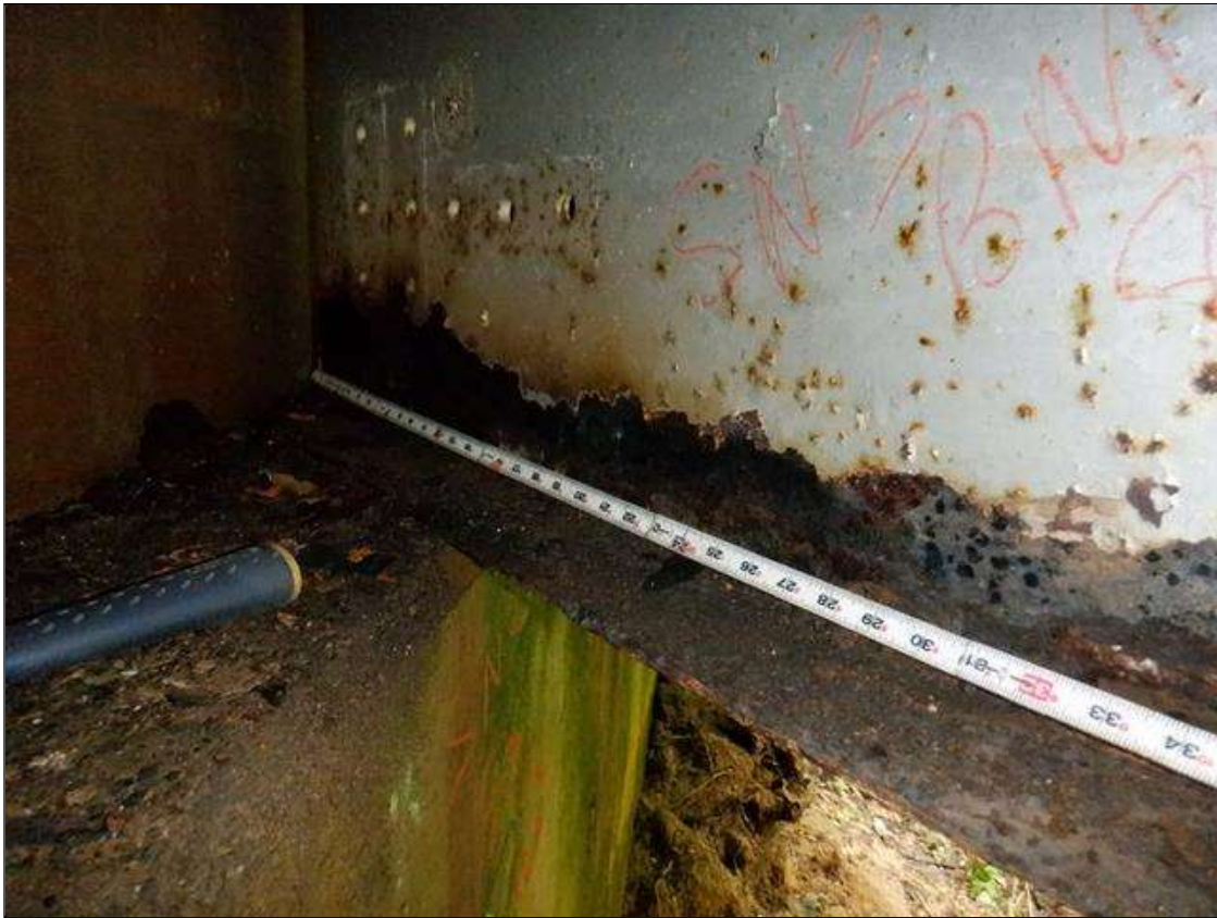
Span 3 Beam 8: [PAR] at far end, active corrosion with section loss; bottom flange [up to 27in x full width - avg rem 3/8in], lower web [up to 7ft x up to 3in - avg rem 5/16in]
