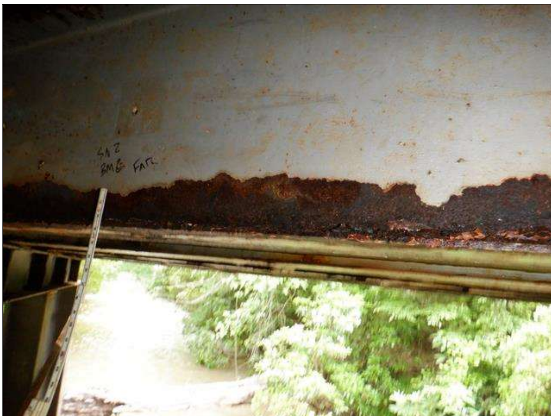
Span 2 Beam 6: [PAR] at far end, active corrosion with section loss; bottom flange [up to 8ft x full width - avg rem 3/8in], lower web [12ft x up to 2in - avg rem 1/4in]
