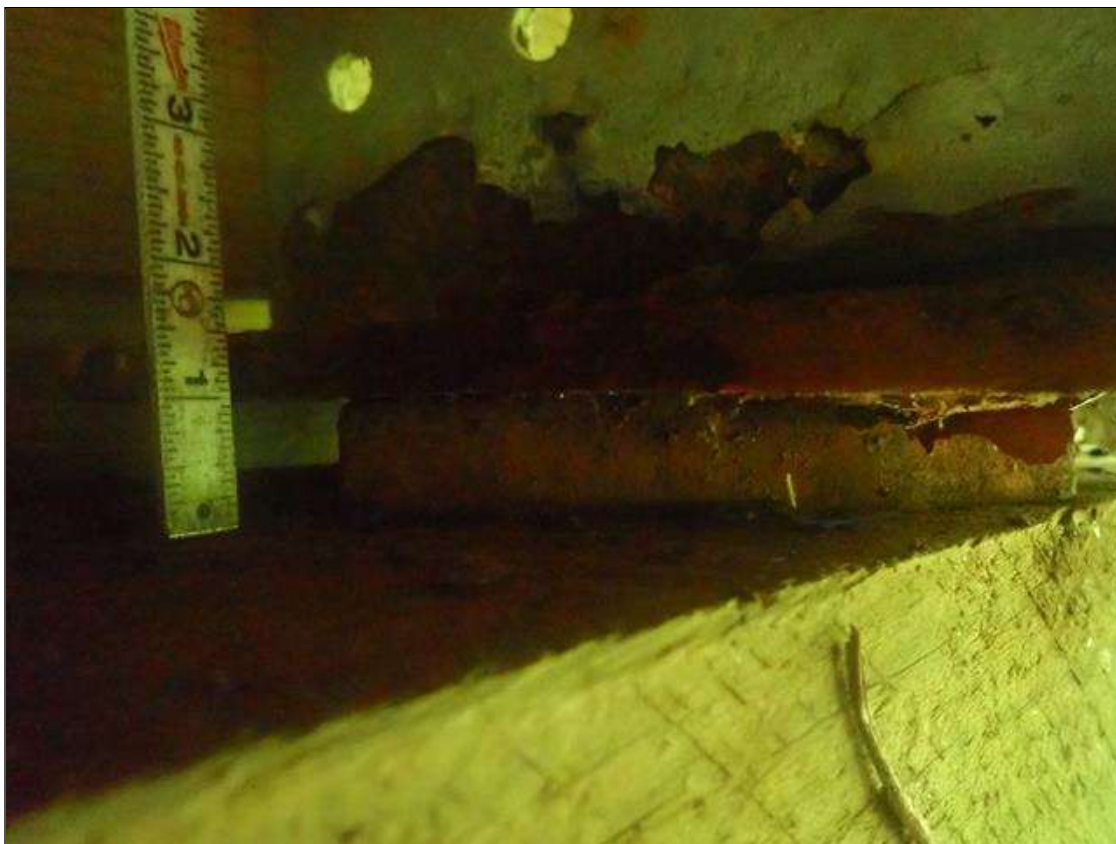
Span 1 Beam 1 Near Bearing: throughout bearing, active surface corrosion [no section loss]
