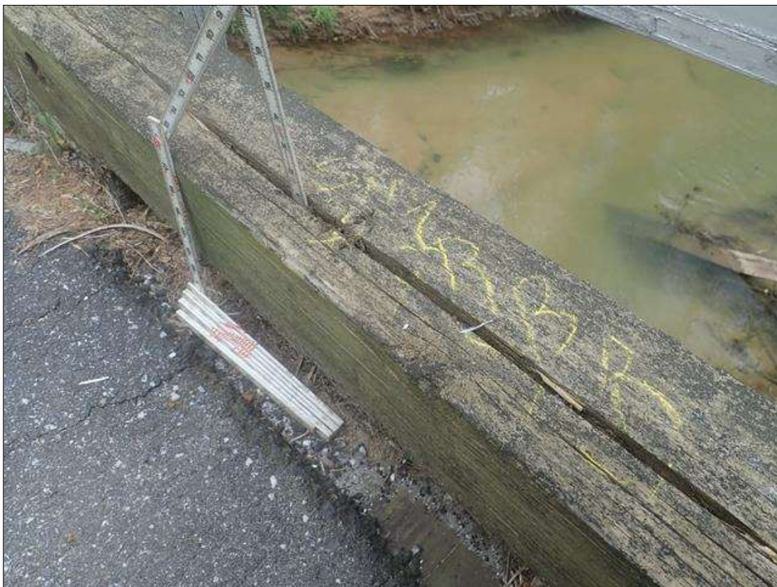
Span 1 Right Bridge Rail: along top of curb, multiple checks [up to 3/8in x up to 1.5in deep]
