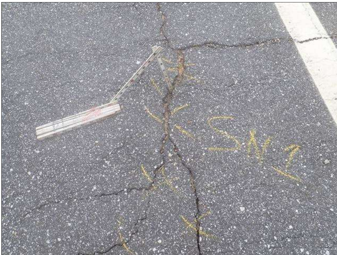
Span 1 Wearing Surface: throughout asphalt wearing surface, multiple transverse cracks and longitudinal cracks [up to full width x up to full length x up to 5/8in]
