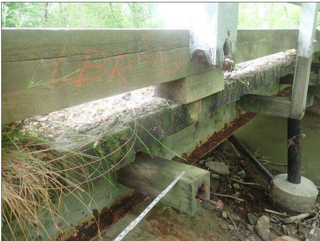
Span 3 Left Bridge Rail: [PAR] at 3rd post from End Bent 2, decay [30in x 100% loss] with missing standoff connection
