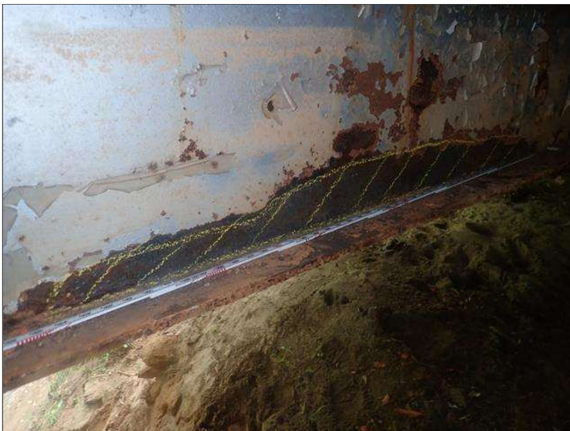
Span 3 Beam 3: [PAR] both sides of lower web 12ft from End Bent 2, active corrosion with section loss [4ft x up to 6in high x 1/4in avg rem]
