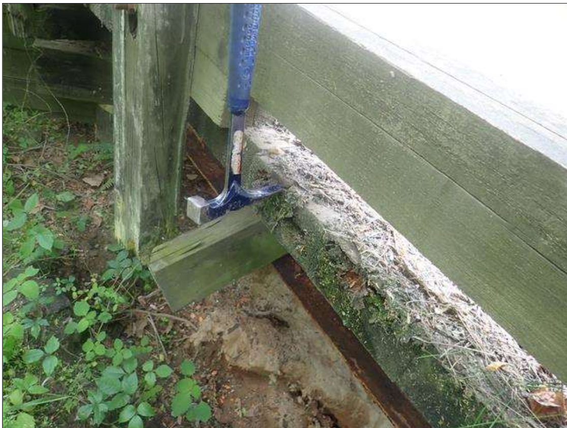
Span 3 Deck: along East and West ends of deck boards, areas of decay/soft timber [less than 10%]
