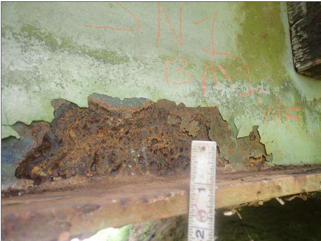
Span 1 Beam 1: along beam, active corrosion with section loss: top flange [full width x 17/32in avg rem], bottom flange [full width x 17/32in avg rem], and lower web [up to 5in high x 11/32in avg rem]
