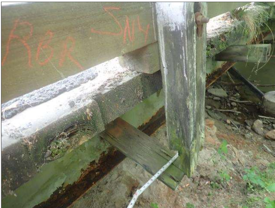
Span 3 Left Bridge Rail: [PAR] at 2rd post from End Bent 2, decay [30in x 100% loss] with missing standoff connection
