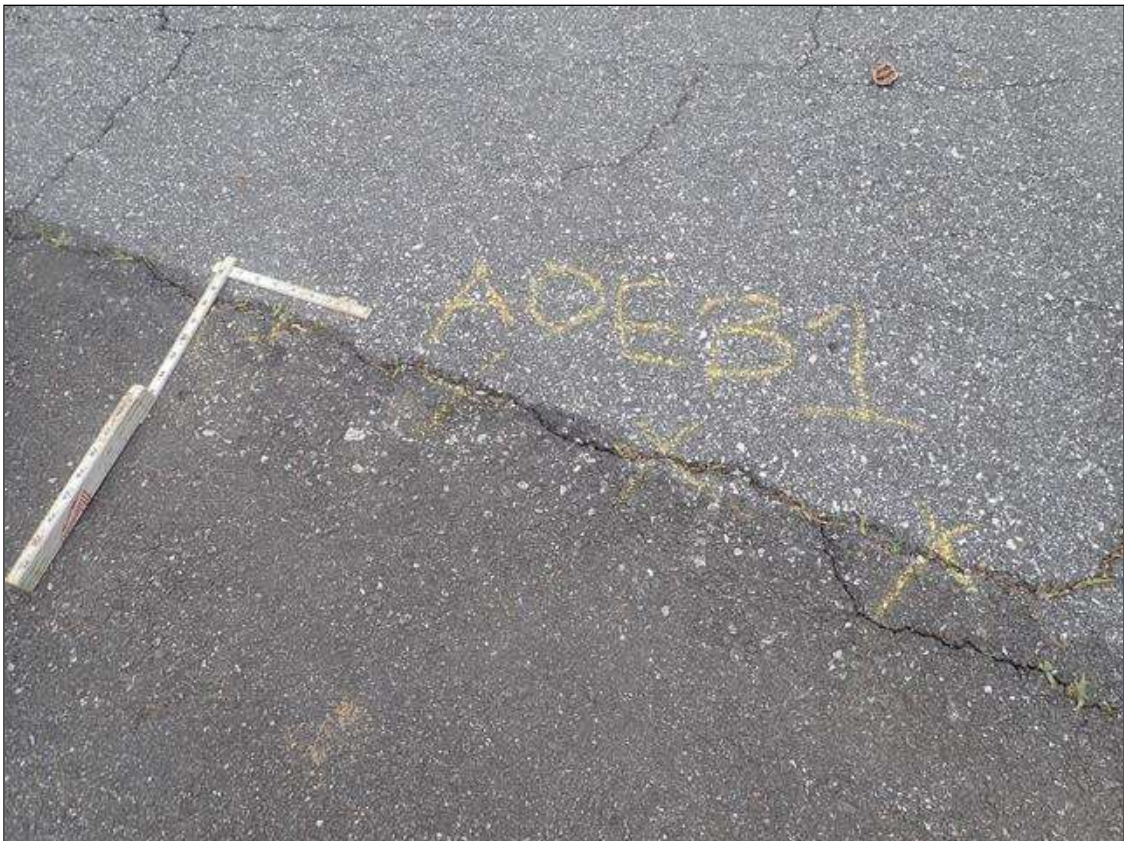
asphalt over end bent 1, transverse crack [full width x up to 3/16in]
