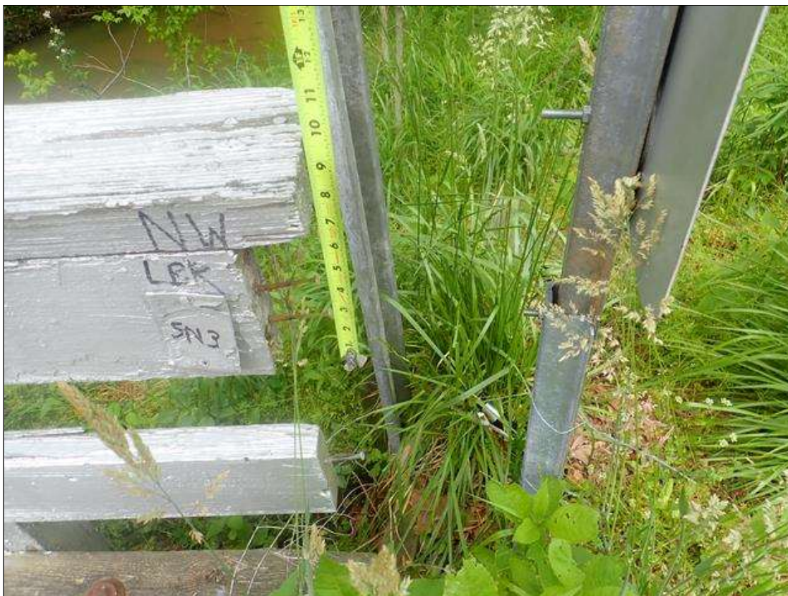
Span 3 Left Bridge Rail: [PAR] at End Bent 2, vertical end board missing
