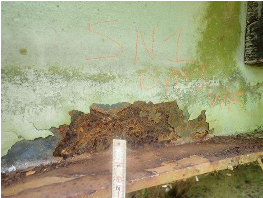
Span 1 Beam 1: along beam, active corrosion with section loss: top flange [full width x 17/32in avg rem], bottom flange [full width x 17/32in avg rem], and lower web [up to 5in high x 11/32in avg rem]
