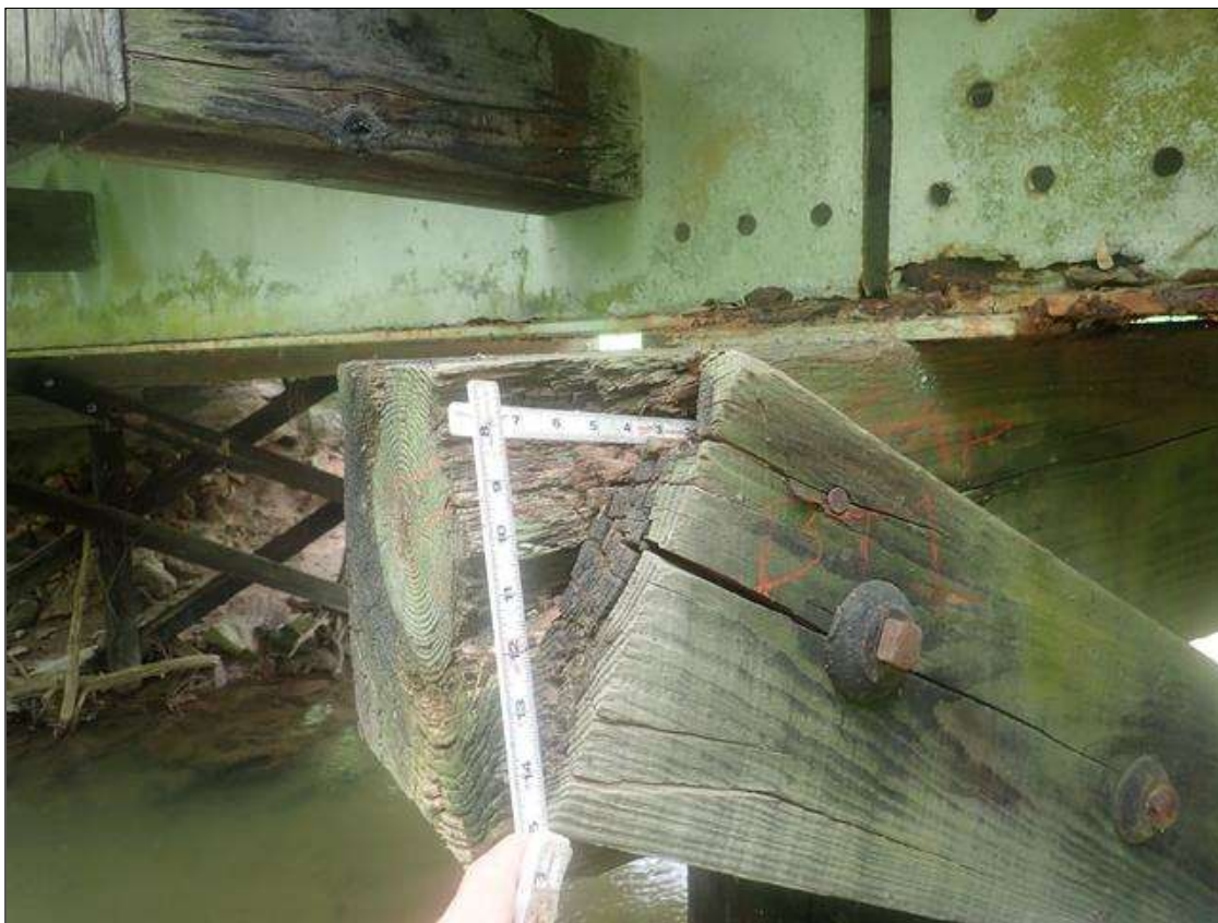
Bent 1 Cap 1: top left corner at West end, decay [9in x 7in x 2in]
