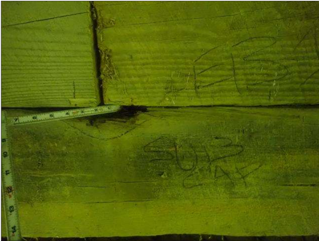
Bent 1 Cap 2: at 4ft from pile 2, decay [6in x 4in x up to 1.5in deep]
