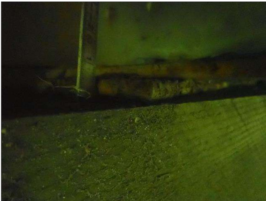
Span 1 Beam 4 Near Bearing: throughout bearing, active corrosion with section loss [up to 1/32in]
