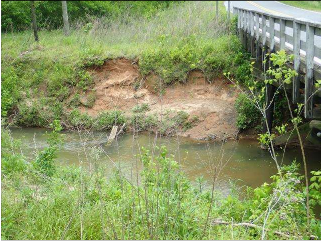
Scour: at both embankments, cut banks [8ft high]
