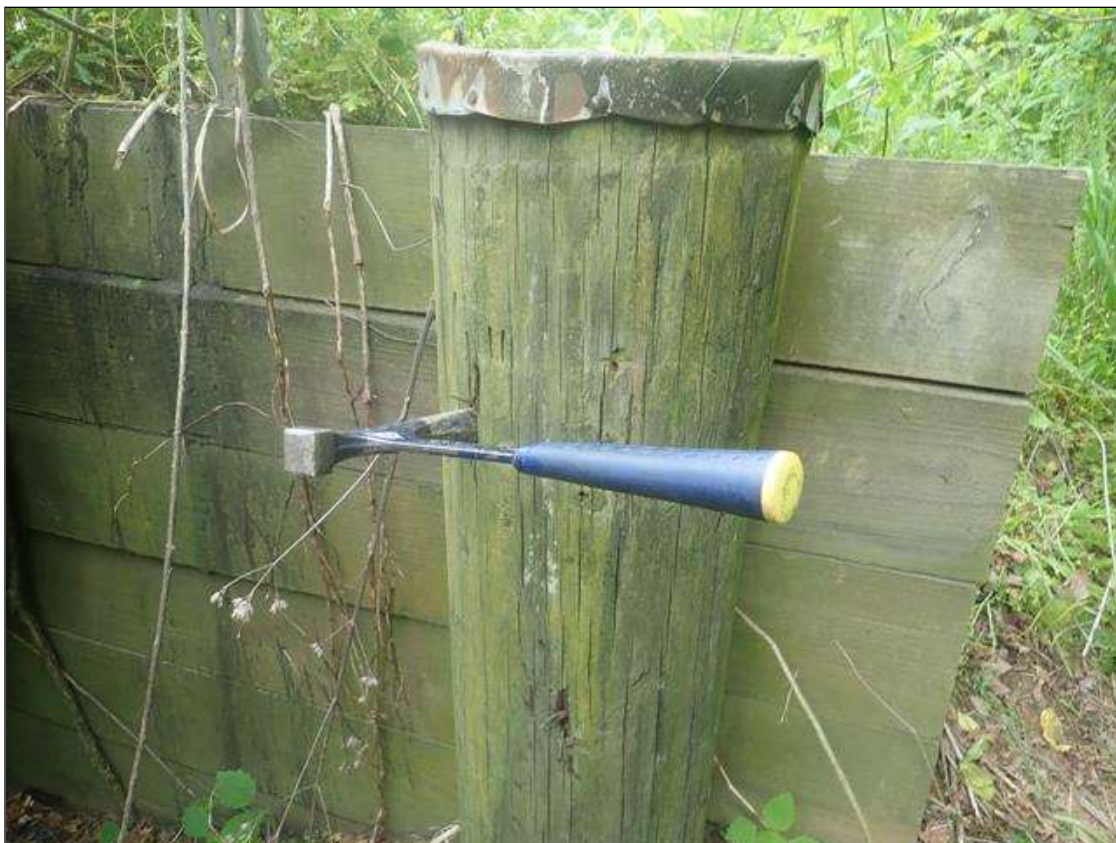
Southwest wingwall along soldier pile around exterior, decay [up to 2in deep] x full circumference
