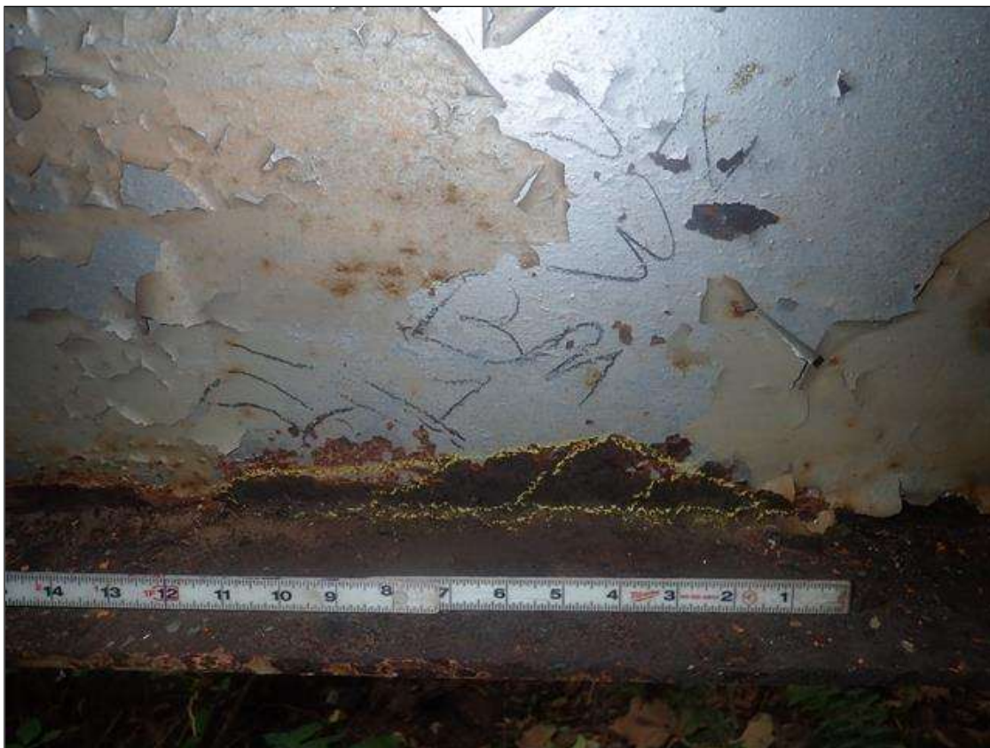
Span 3 Beam 1: [PAR] lower web at 3ft from End Bent 2, active corrosion with section loss [1in x up to 2in high x 3/16in avg rem]
