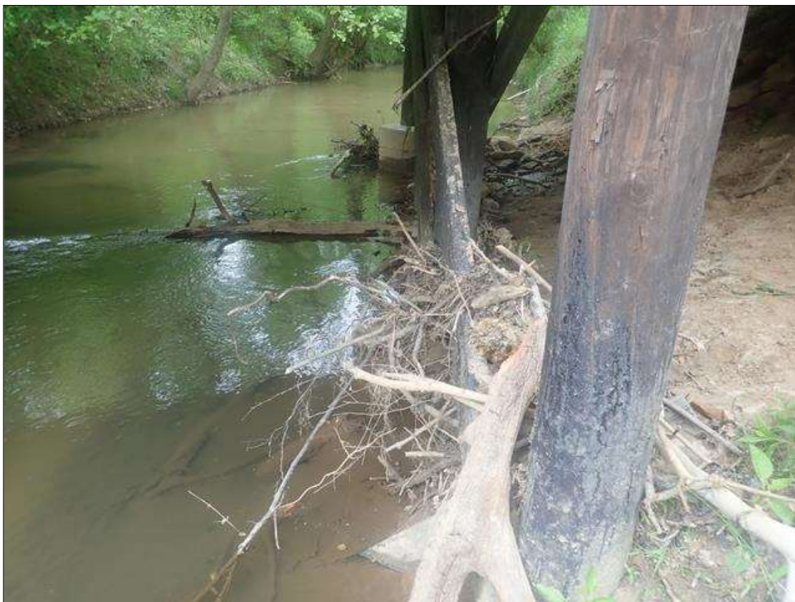
At bent 2 piles, drift accumulation [up to 6in]
