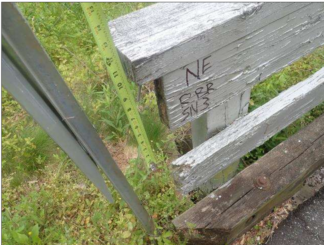
Span 3 Right Bridge Rail: [PAR] at End Bent 2, vertical end board missing
