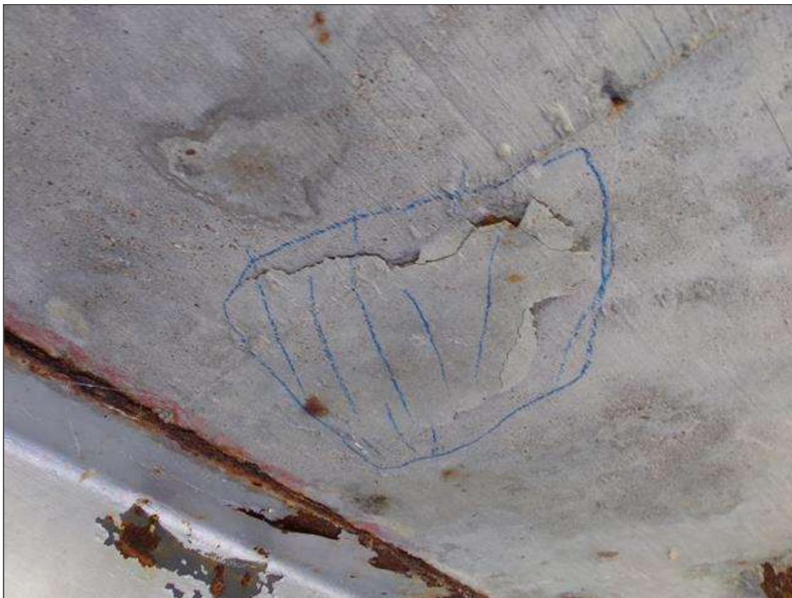
Span 3 Deck: 7" diameter area of delamination on south overhang at 2' from pier 2
