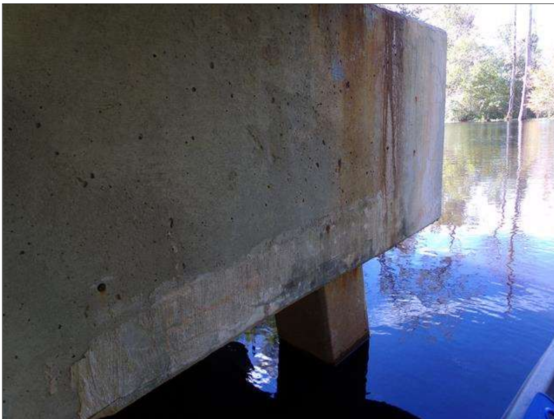
Bent 2 Cap 1: 5ft x up to full height sound patched area with hairline map cracking on west face at south end.
