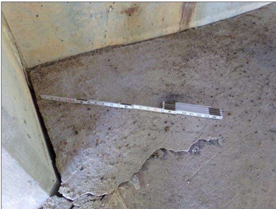
Slope Protection: End bent 1 slope protection 3' long x 2' wide area of delamination on front of slope in bay 3 at brace pile cap
