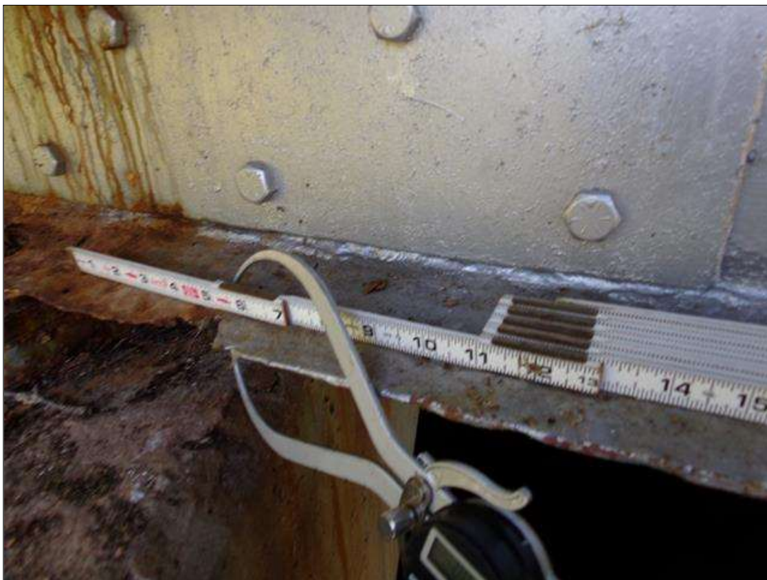
Span 3 Beam 4: PM---2' long x full width x down to knife edge area of advanced section loss (0.20" average thickness remaining) on bottom flange at pier 2. 5" long x 1" wide area of 100% section loss on north bottom flange. Previously cleaned and painted with rust staining reactivated.
