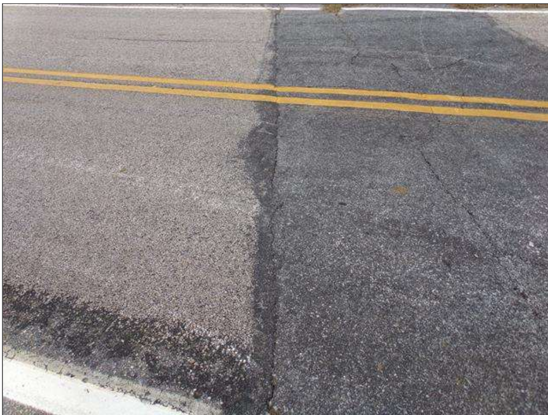
Span 3 Wearing Surface: Full width transverse crack up to 1/4" wide over abutment.
