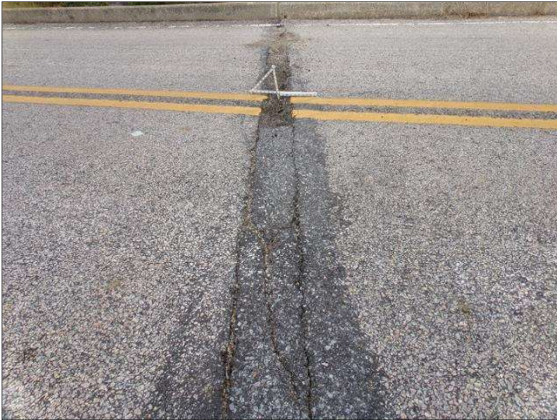
Span 1 Wearing Surface: PM--12' long pothole starting at center line out in westbound travel lane over pier 1 up to 6" wide x 2" deep full width of bridge. Pothole is full of gravel 1" deep.
