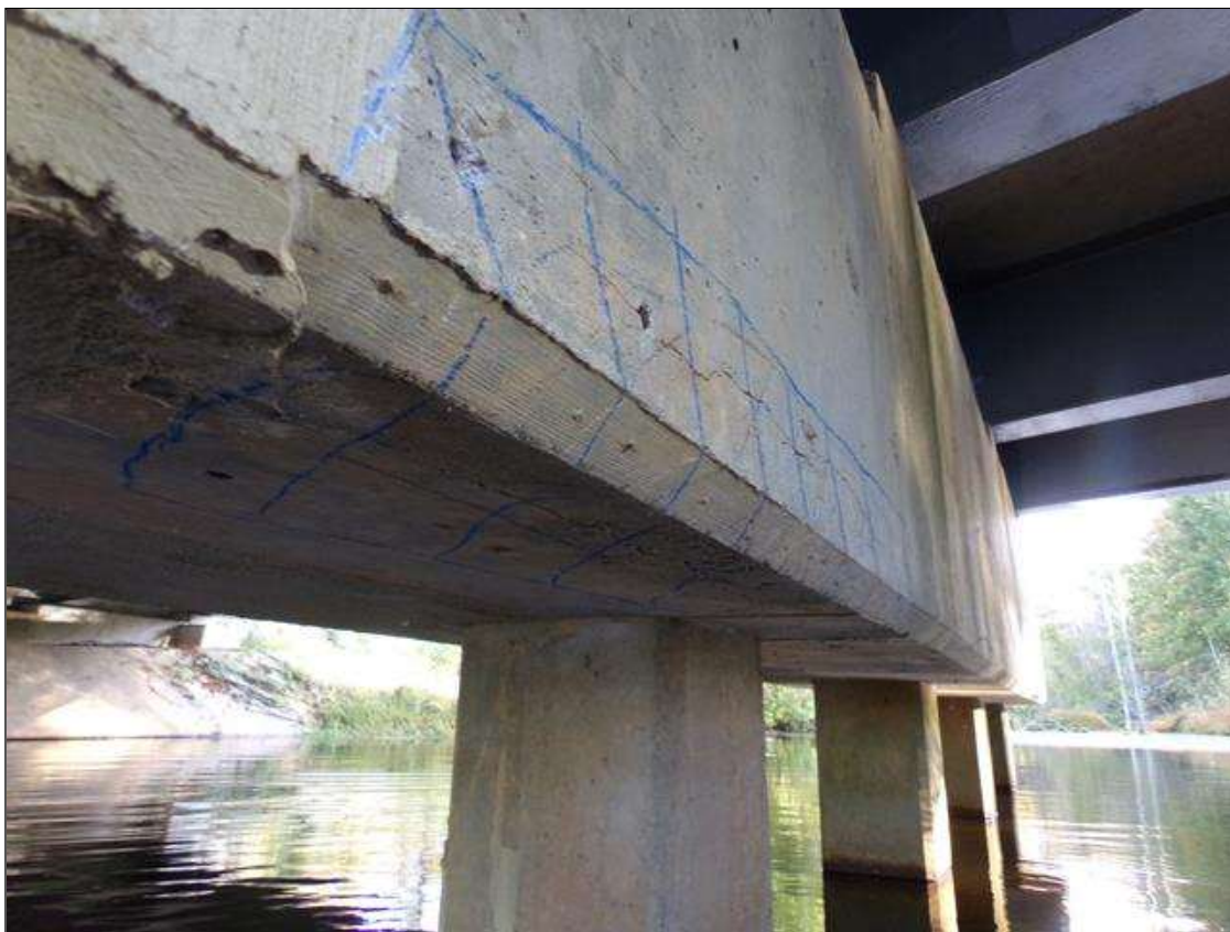
Bent 1 Cap 1: 3' long x 4" high x 1' wide area of delamination on bottom of east face of cap between piles 4 and 5
