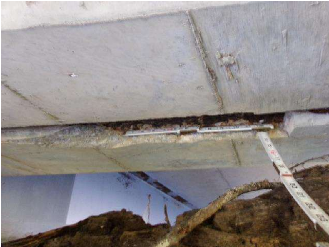
End Diaphragm: Span 3 2' long x 3" wide x 3" d spall with exposed rebar with no measurable section on bottom west face corner
