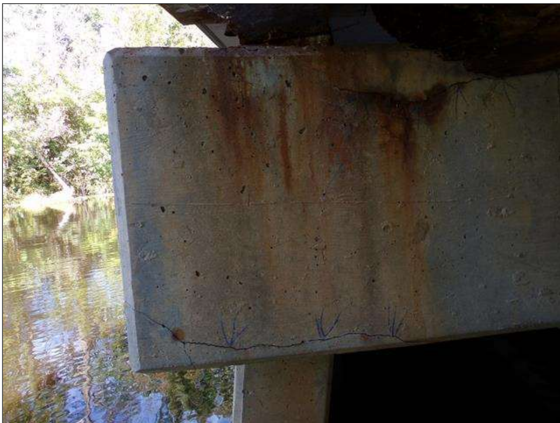
Bent 2 Cap 1: 3' long x up to 1/8" wide horizontal crack with rust staining on south end at bottom of cap that wraps around 3" on south end
