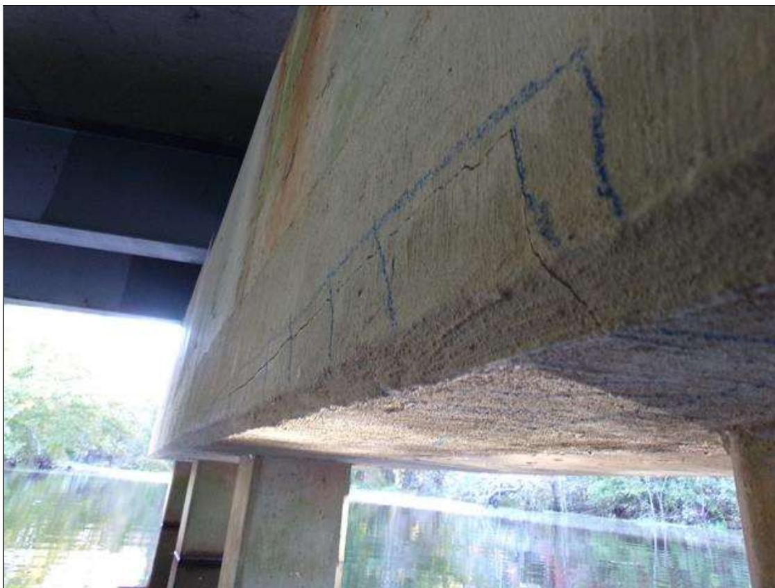
Bent 1 Cap 1: 3' long x 3" high x 1' wide area of delamination on bottom of west face of cap at pile 4
