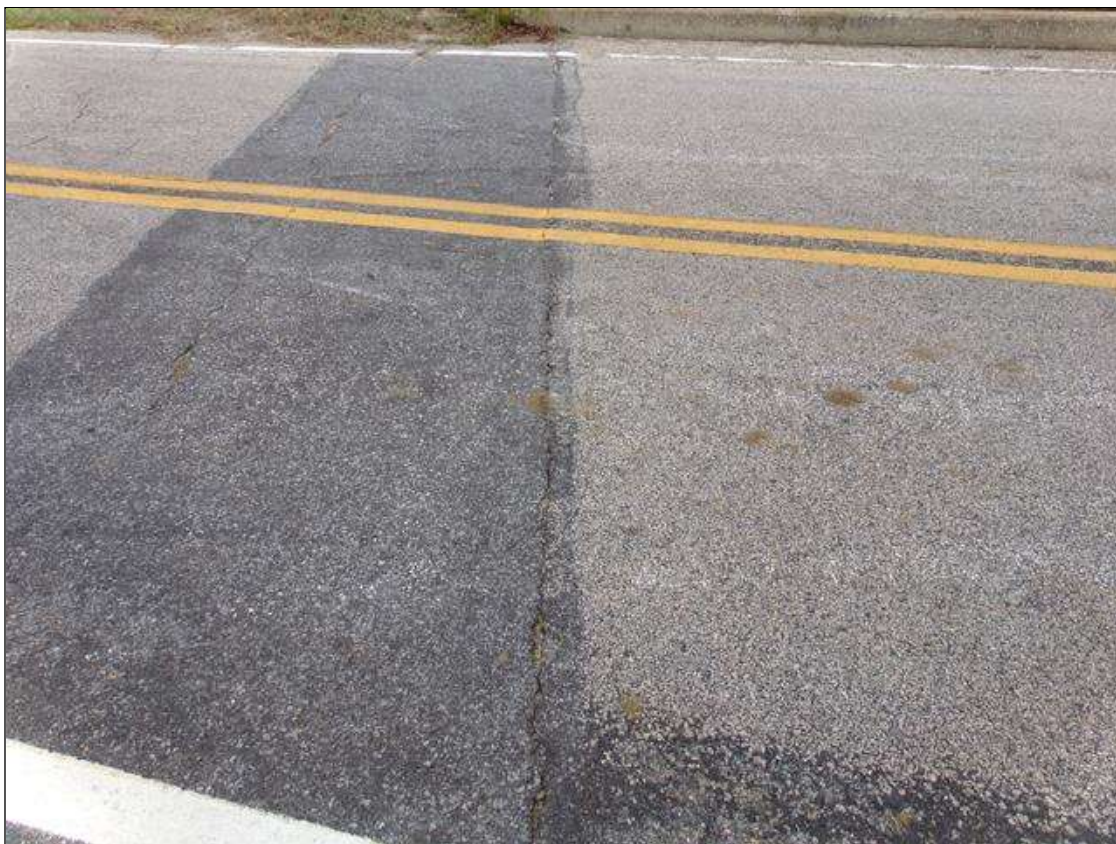
Span 1 Wearing Surface: Full width transverse crack up to 1/4" wide over abutment.
