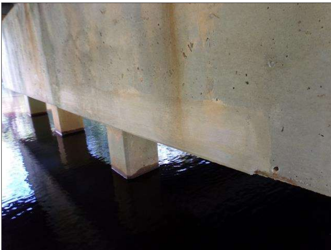
Bent 2 Cap 1: 5' long x 6" high sound patched area starting at pile 3 extending out to pile 4 on west face
