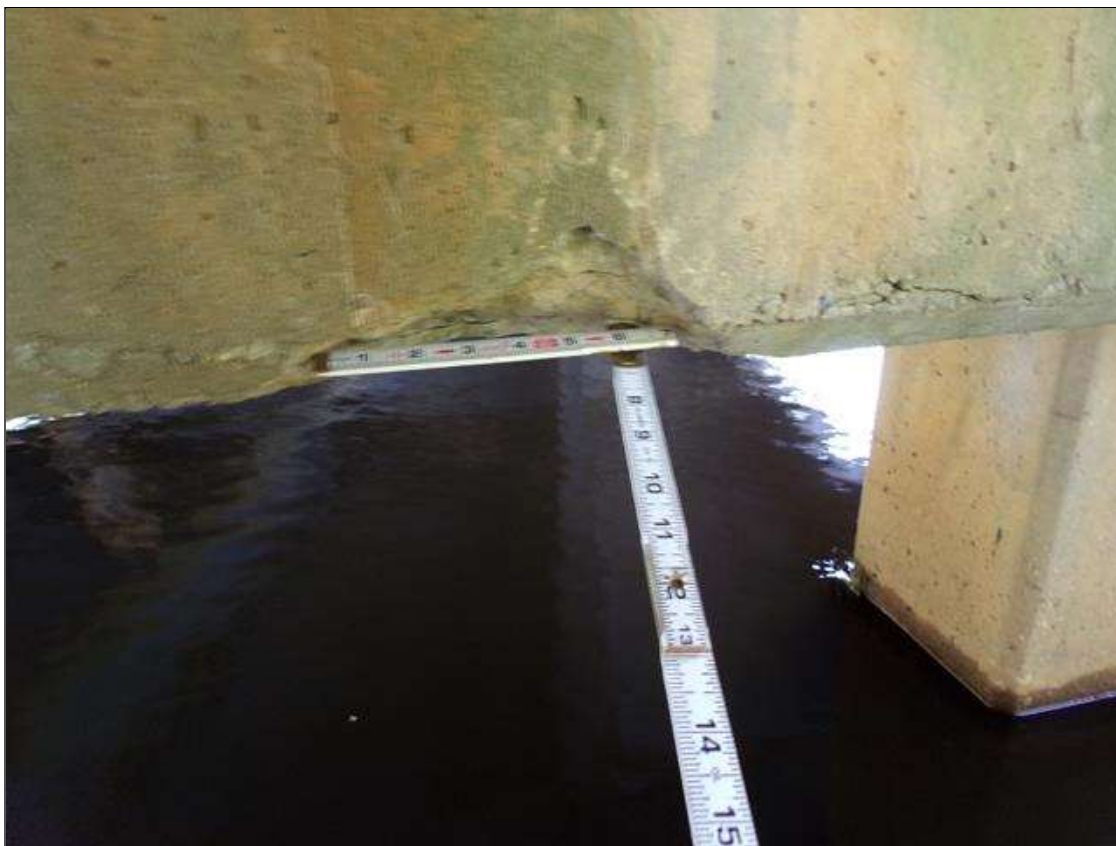
Bent 2 Cap 1: 8" long x 7" high x 3" deep spall with no exposed rebar between piles 2 and 3 on bottom of east face of cap
