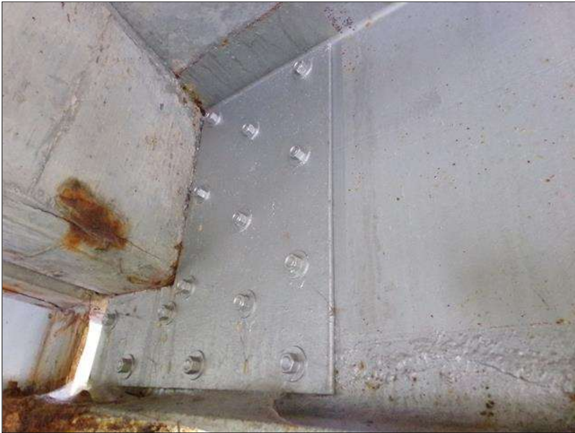
Span 1 Beam 4: 2' high x 2' long x 3/8" thick steel plate added over pier 1 on both faces of web
