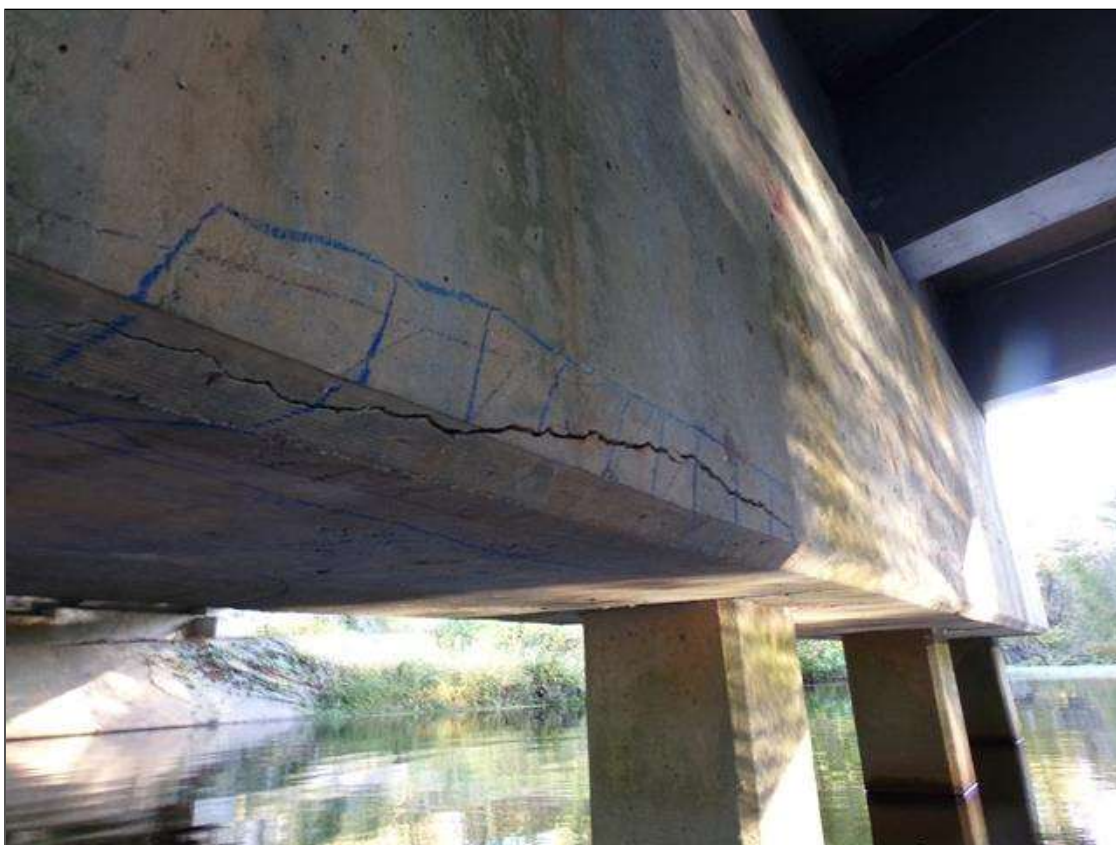
Bent 1 Cap 1: 2.5' long x 3" high x 4" wide area of delamination on bottom of east face of cap between piles 3 and 4
