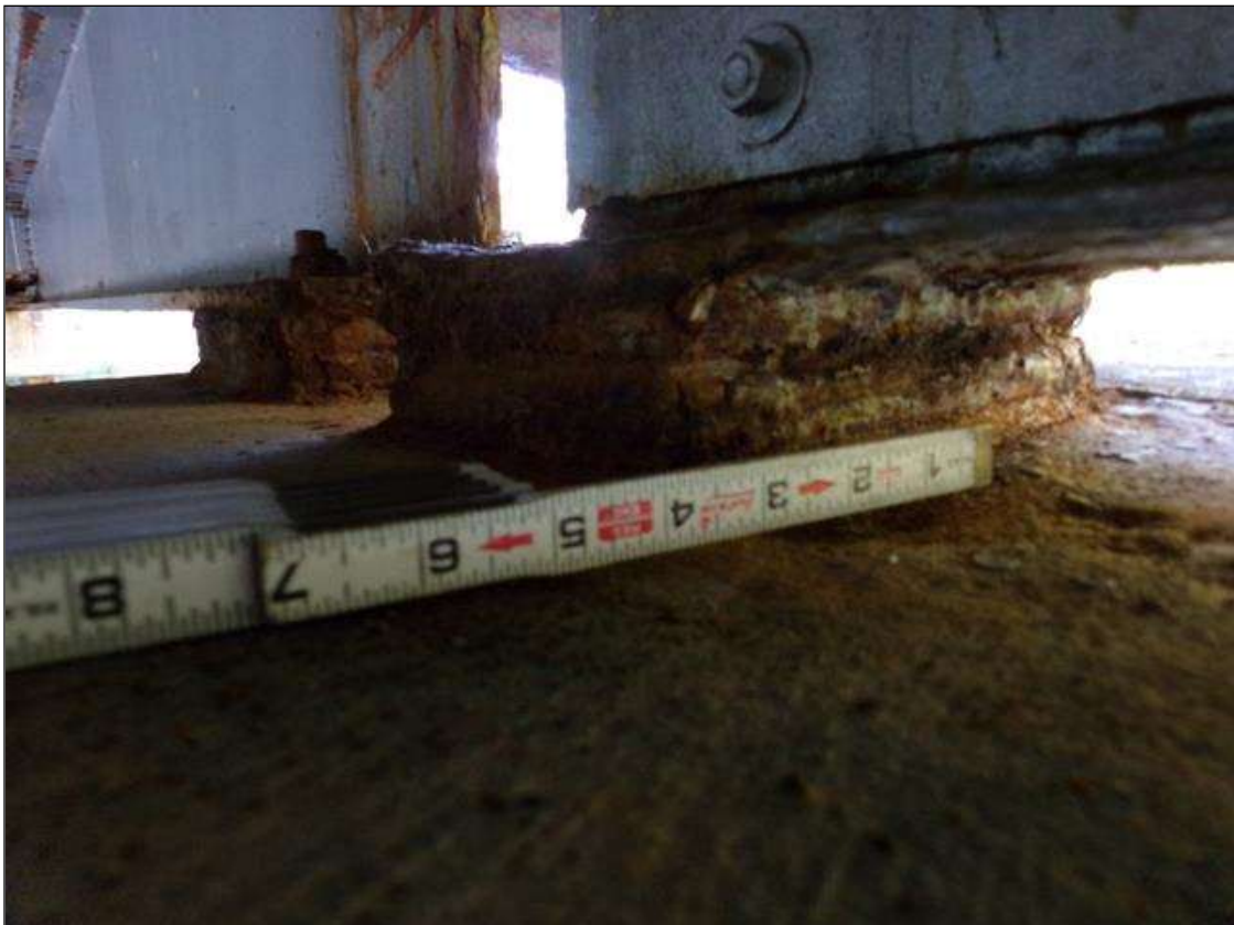
Span 1 Beam 4 Far Bearing: Previously cleaned and painted, but corrosion has reactivated with no additional section loss (up to 1/8") and anchor bolt nut corroded (100%)
