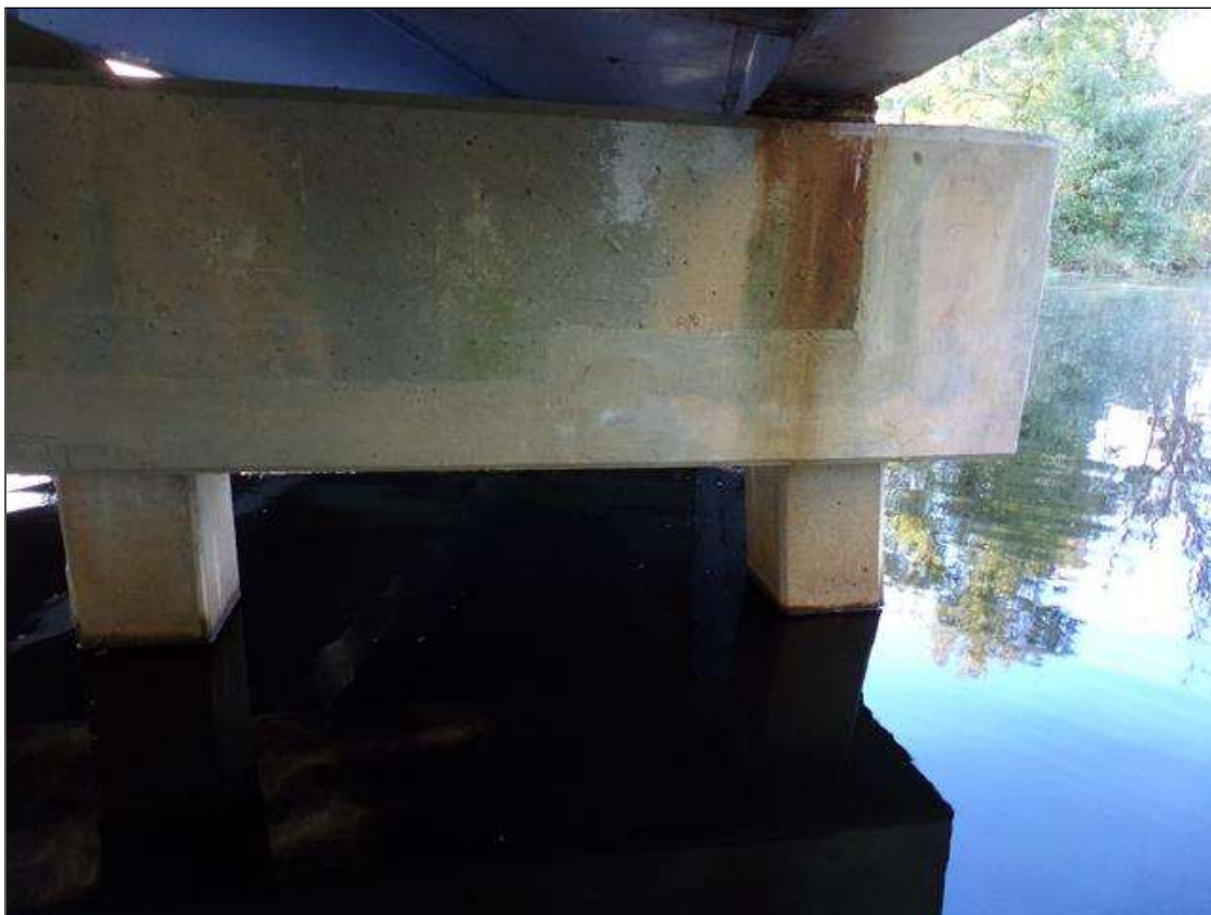
Bent 1 Cap 1: 7' long x up to full height sound patched area on west face of cap starting at pile 4 and extending to south end of cap
