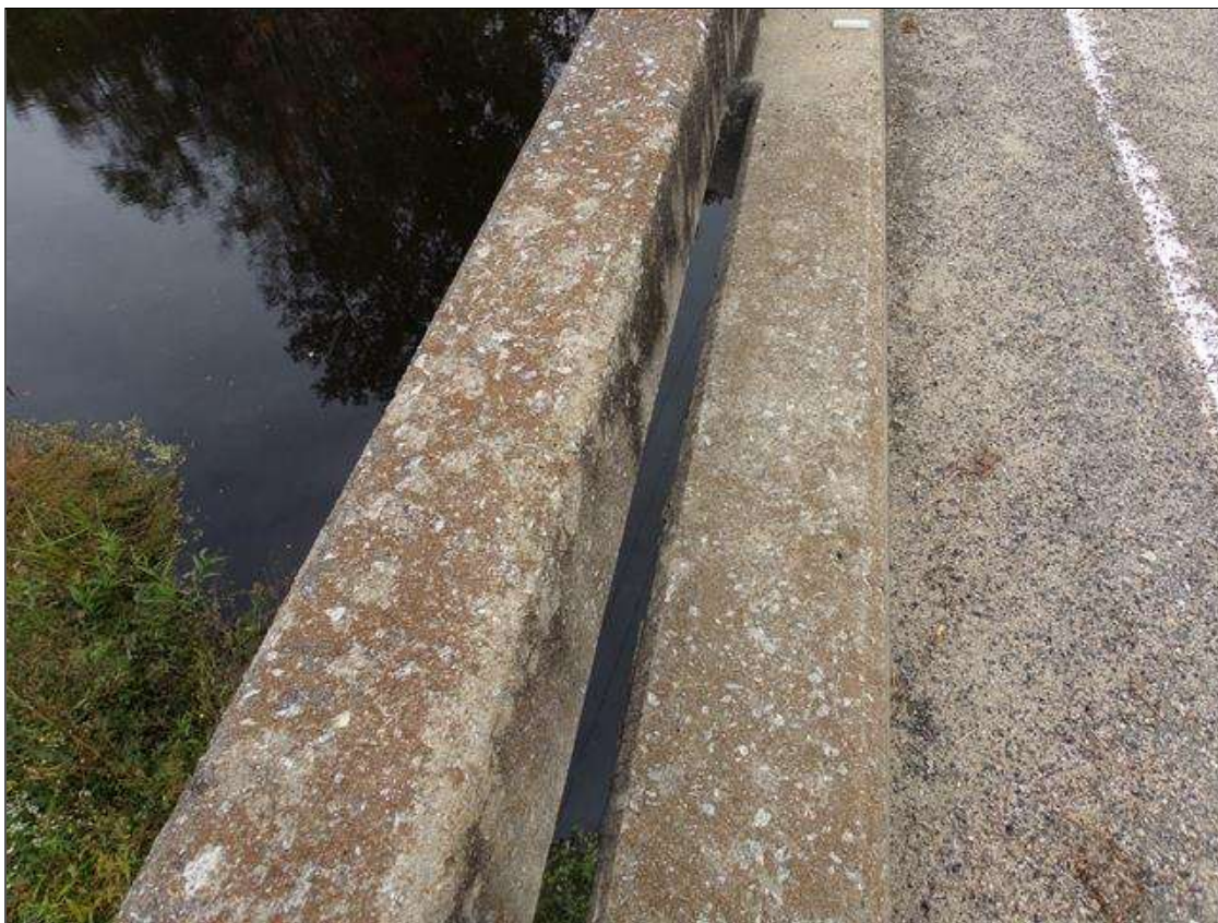
Typical top rail and parapet, scaling with exposed aggregate (full length x full width), left rail span 1 shown, right rail similar.
