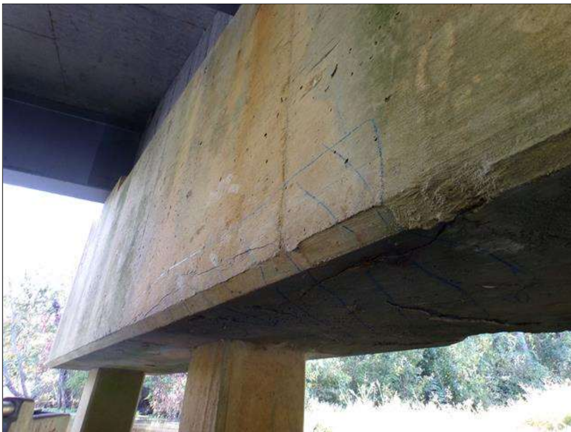
Bent 2 Cap 1: 3.5' long x 6" high x full width on bottom of cap on west face under beam 2
