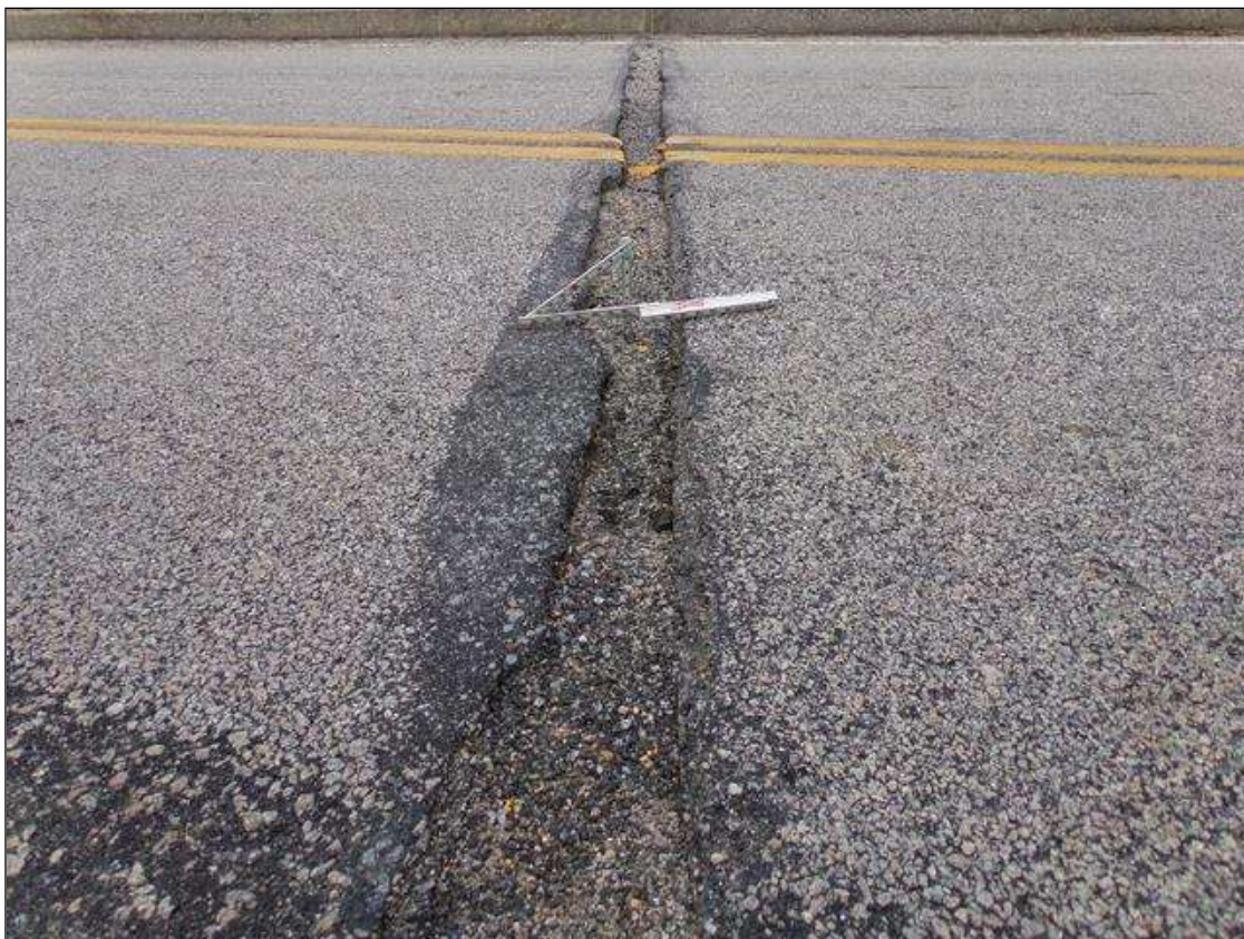
Span 2 Wearing Surface: PM--Full width pothole over pier 2 up to 6" wide x 2" deep full width of bridge. Pothole is full of gravel 1" deep.
