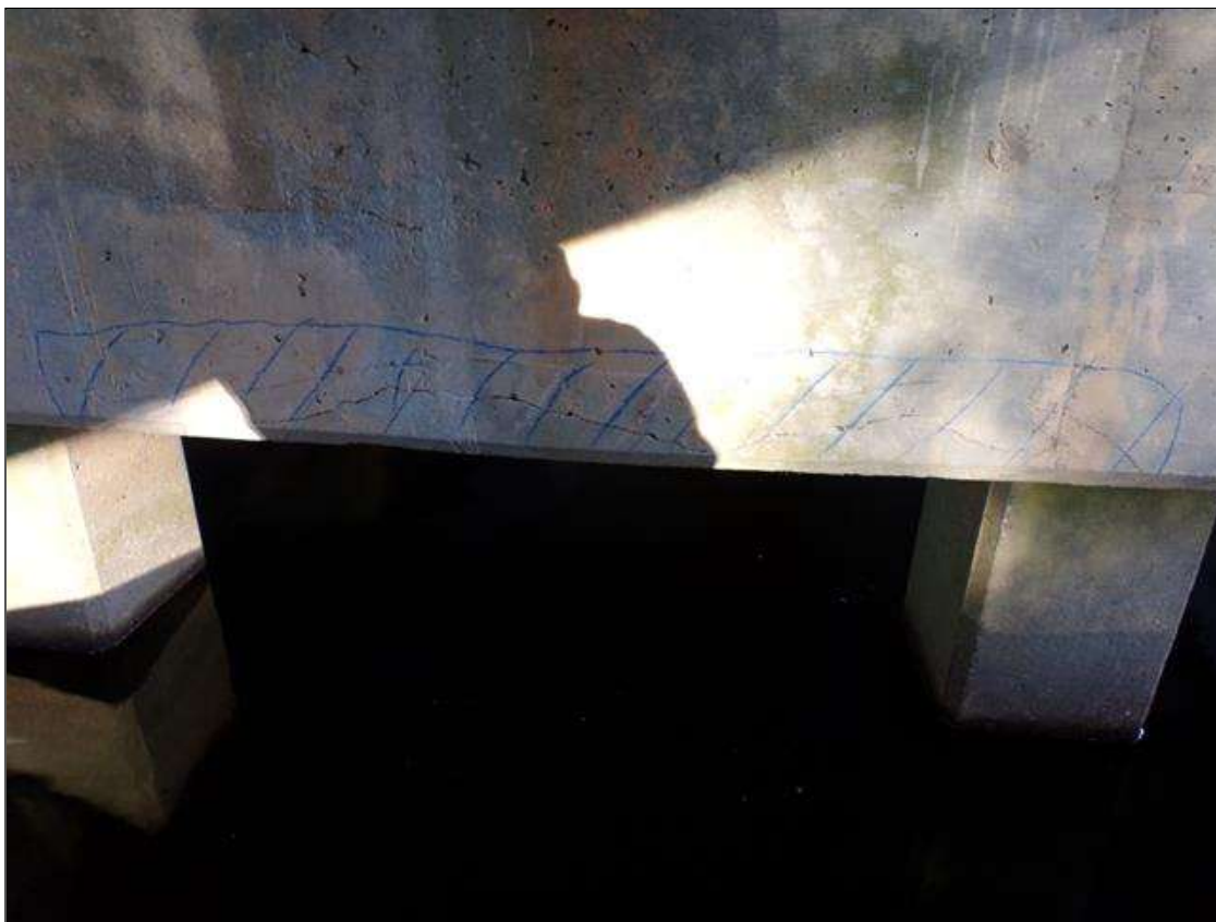
Bent 1 Cap 1: 3.5' long x 5" high area of delamination on bottom of east face of cap between piles 2 & 3
