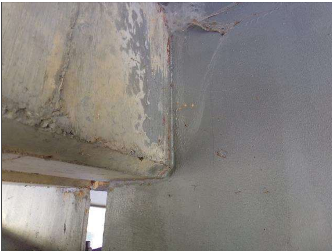
Span 1 Beam 2: Typical painted over pitting (1' long x 1" wide x up to 1/8" deep) at interface with concrete end diaphragms at piers.
