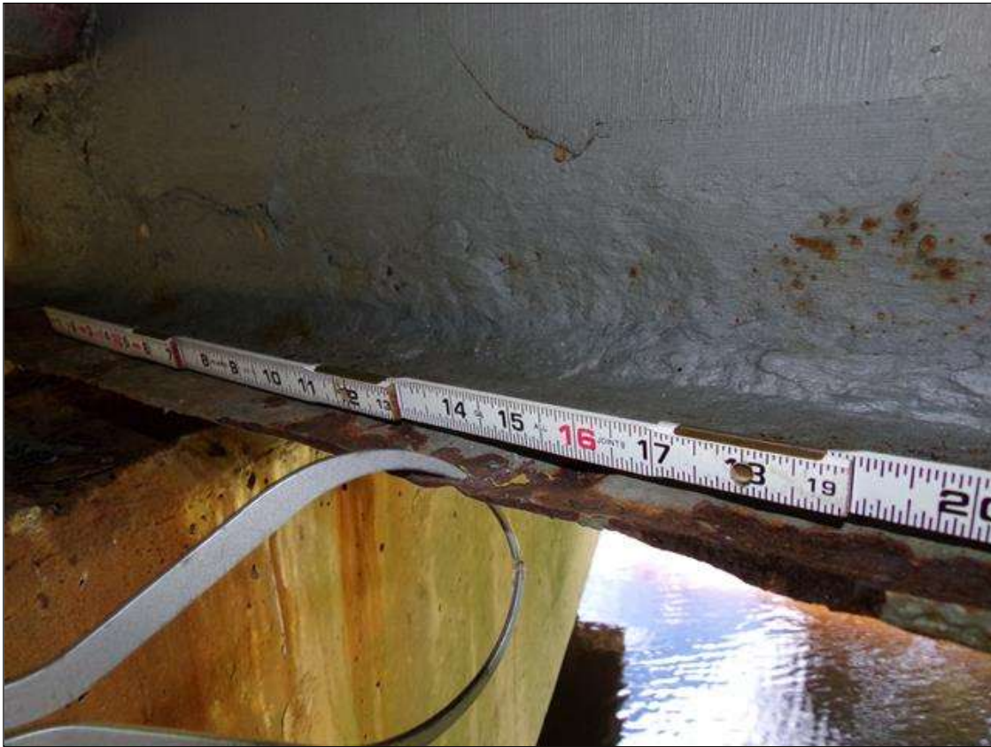
Span 3 Beam 2: PM---2' long x full width x down to knife edge area of advanced section loss (0.33" average thickness remaining) on bottom flange at pier 2. 1.5" long x 3/4" wide area of 100% section loss on south bottom flange at 16" from bearing. Previously cleaned and painted with rust staining reactivated.
