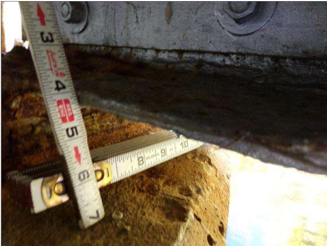
Span 1 Beam 4: 1' long painted over corrosion with section loss (3/8" remaining thickness) on outer edges (2") of bottom flange with 7/16" average remaining thickness across full width. 11/16" original thickness.
