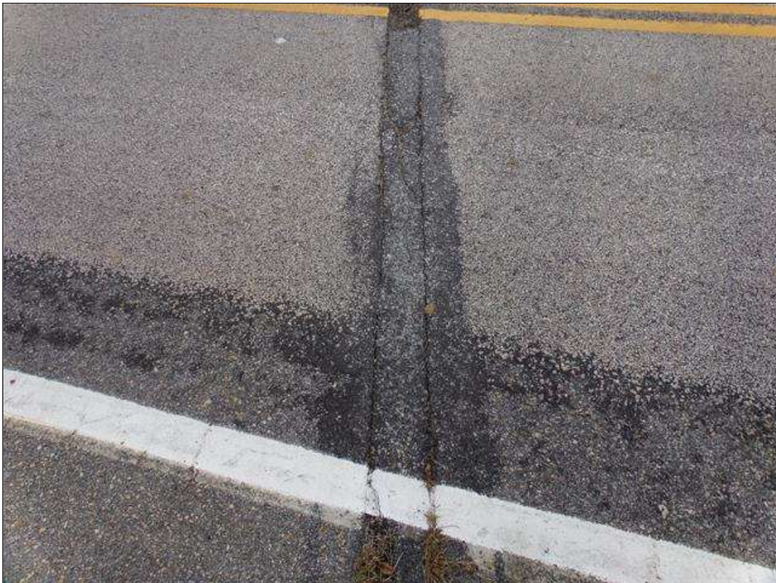
Span 1 Wearing Surface: Eastbound travel lane and both shoulders over end bent 1 have 2 transverse cracks up to 1/4" over pier 1.
