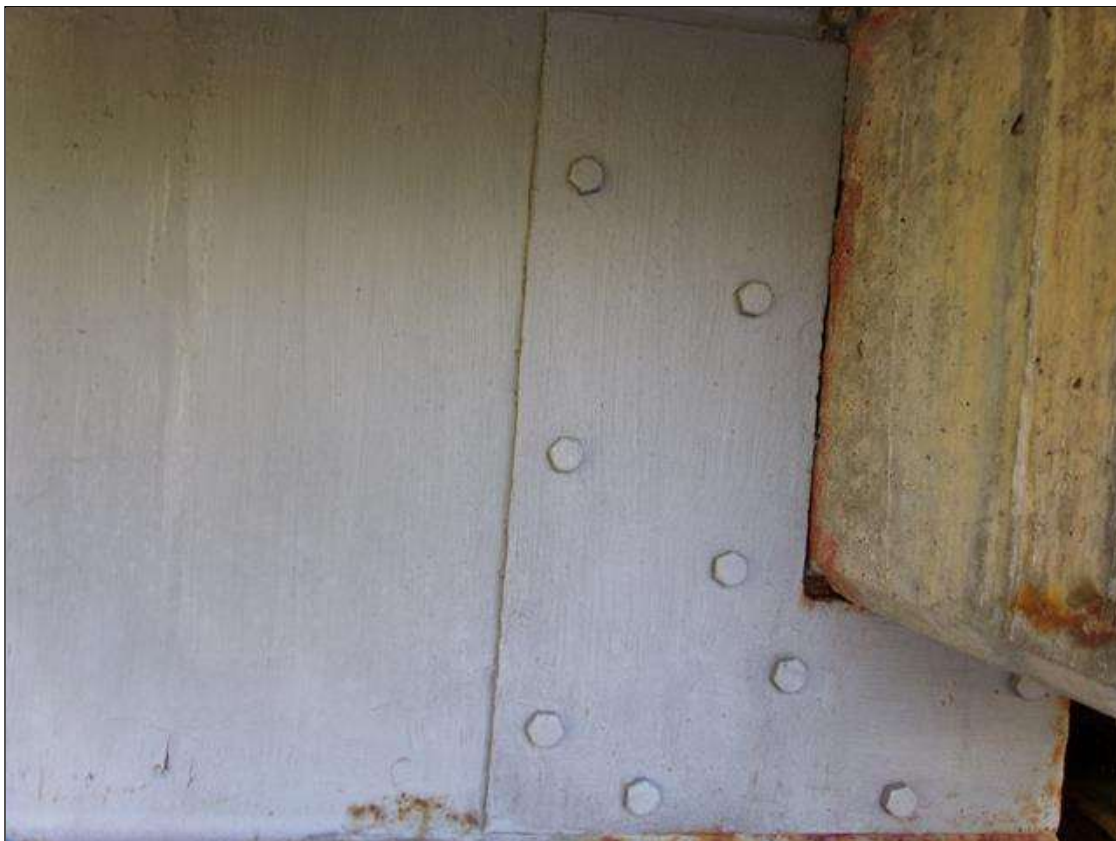
18" long x 20" long added at end of beam 4 at pier 2 span 2
