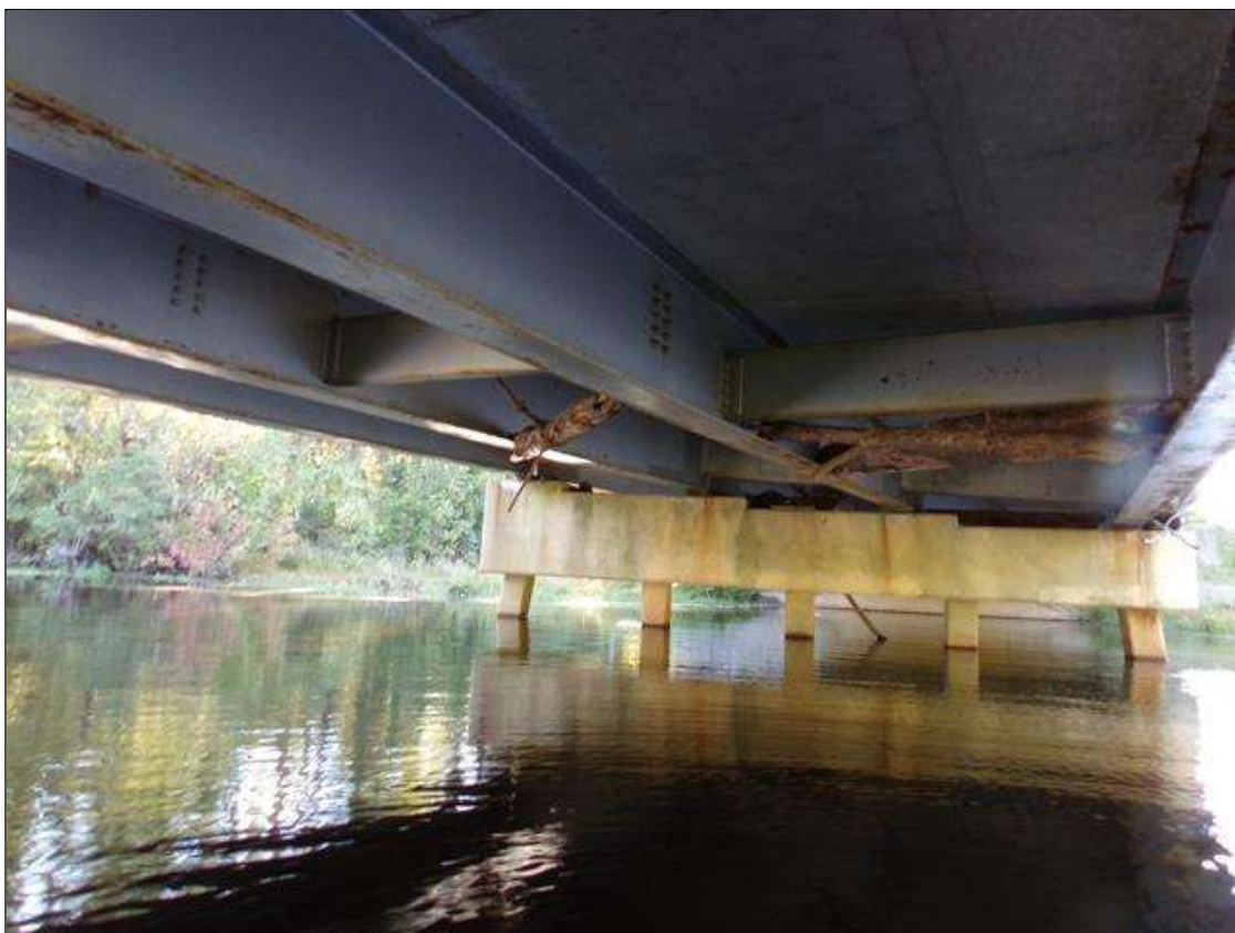
Drift accumulation between beams in bays 2 and 3 in span 2 and on top of pier 2 cap within all bays and south end
