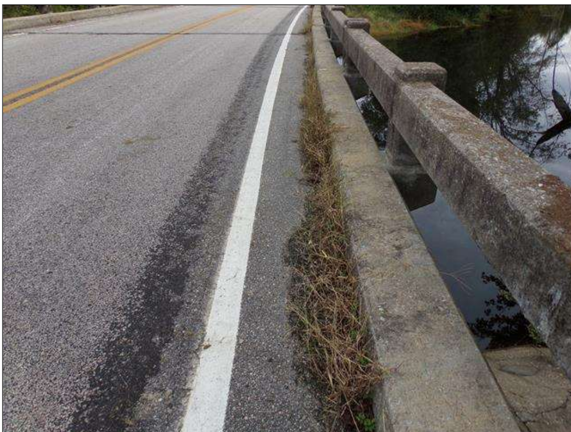
Debris accumulation with vegetation growth entire length of right rail 10" wide with a few drains partially blocked.
