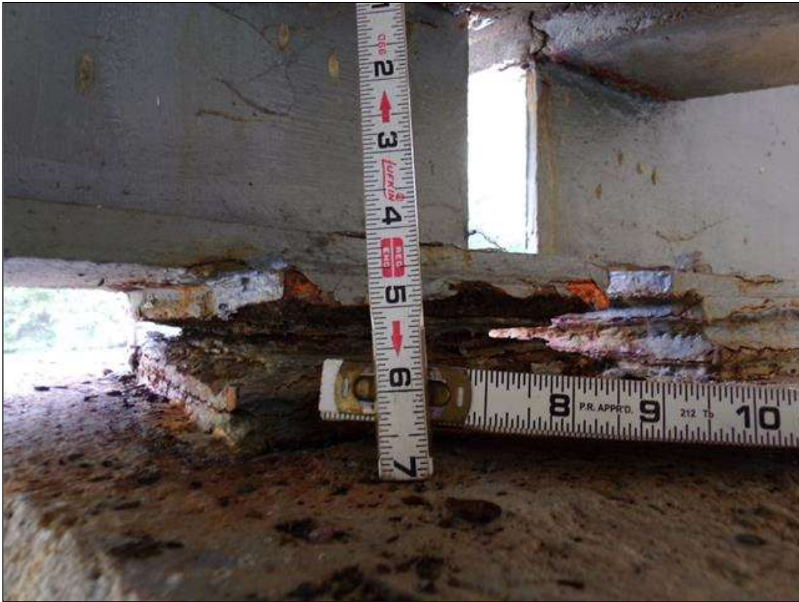
Span 2 Beam 1 Far Bearing: PM---Previously cleaned and painted over section loss (approximately 40%) with reactivated corrosion with nearly 60% section remaining.
