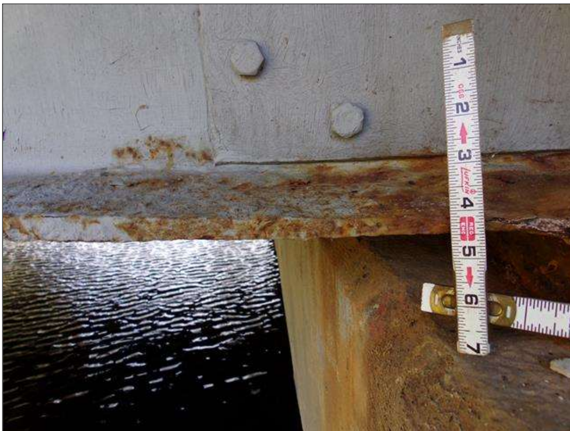
Span 2 Beam 4: bottom flange at bent 2, pitting (1ft x 5in) (0.30in avg rem) (recently cleaned and painted with rust staining)
