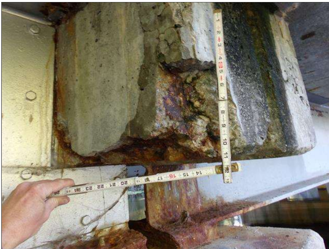
End Diaphragm: Full height x full width x up to 3" deep area of delamination/spall on southwest corner on south overhang in span 1
