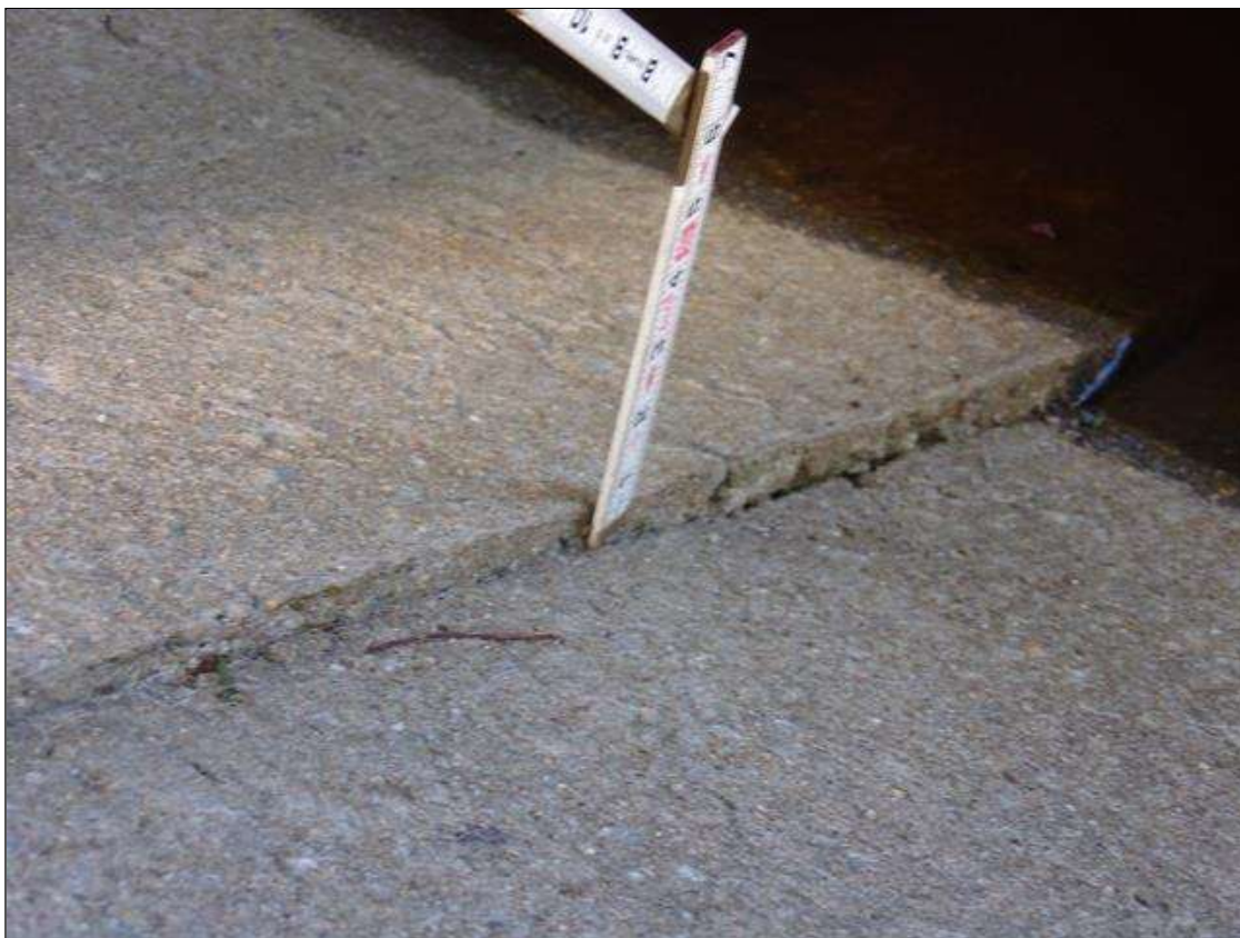
Slope Protection: End bent 1 slope protection south end at waterline is settled for 2.5' long x up 1" deep
