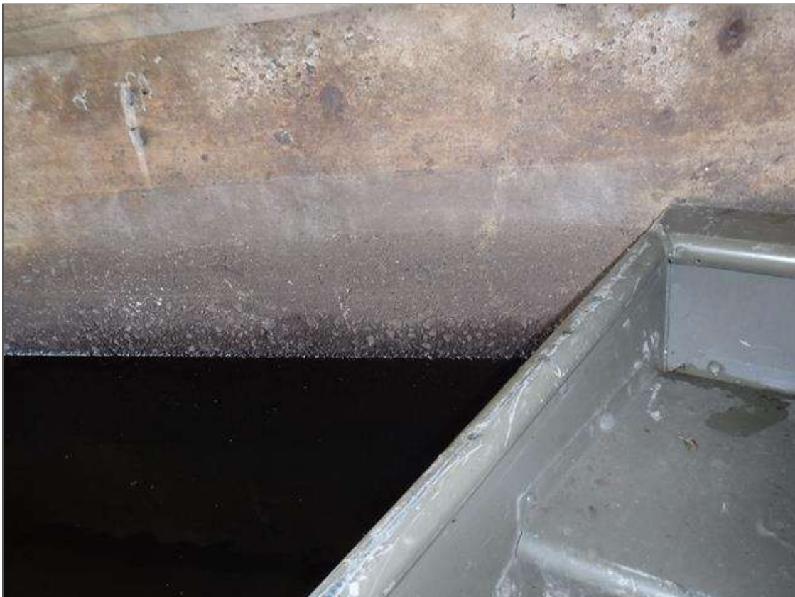
ABRASION IN FACE OF CAP BENT 1
