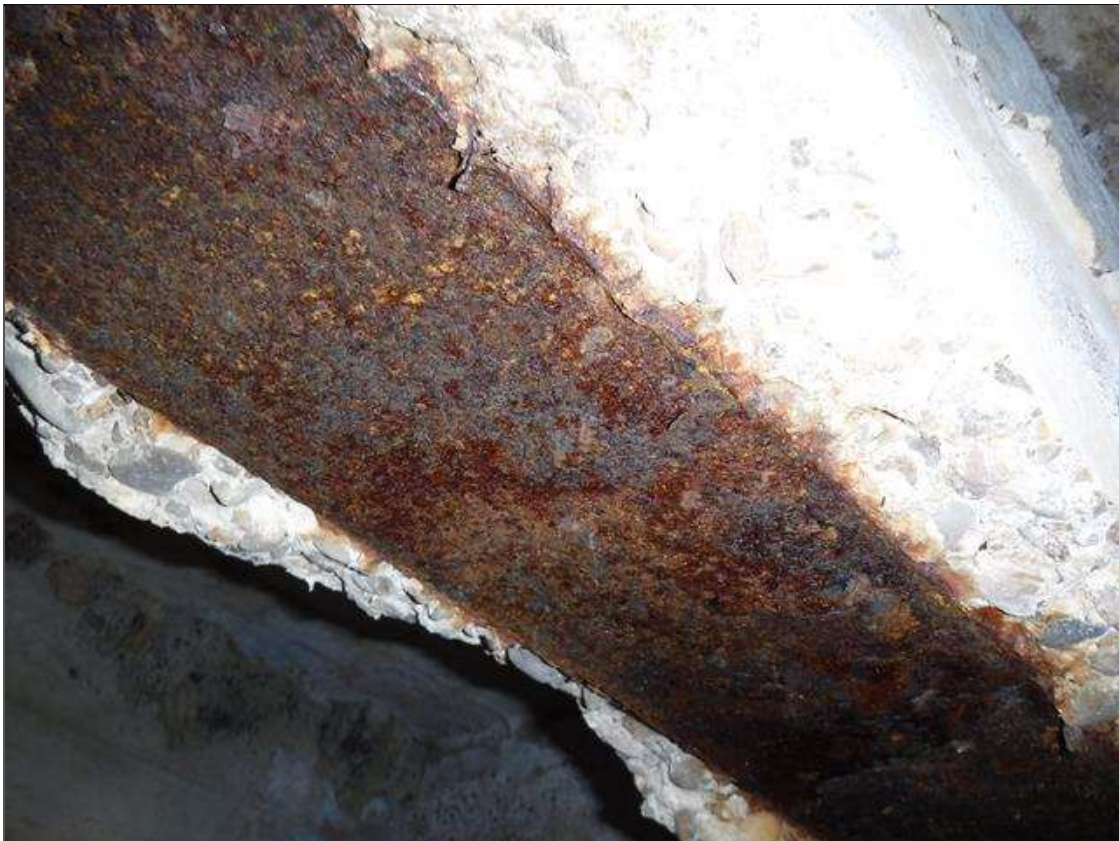
Span 2 Beam 4: RUSTY BOTTOM OF BEAM AT BENT 1
