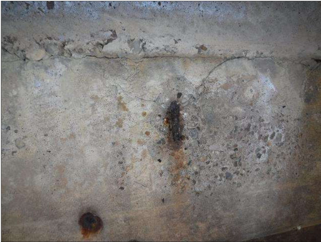
Bent 1 Cap 1: SURFACE SPALLS IN FACE OF CAP
