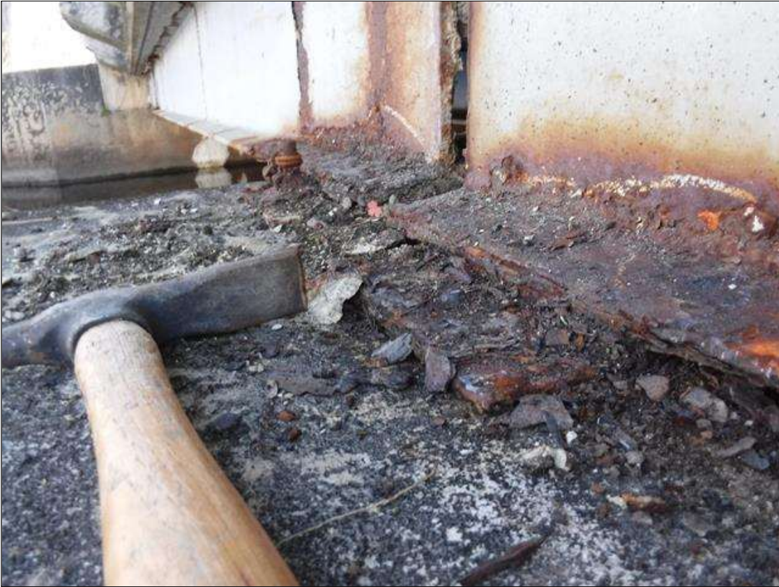
Span 1 Beam 1 Far Bearing: MISSING ANCHOR BOLT BEAM 1 BEARING OVER BENT 1 PRIORITY MAINTENANCE ISSUED
