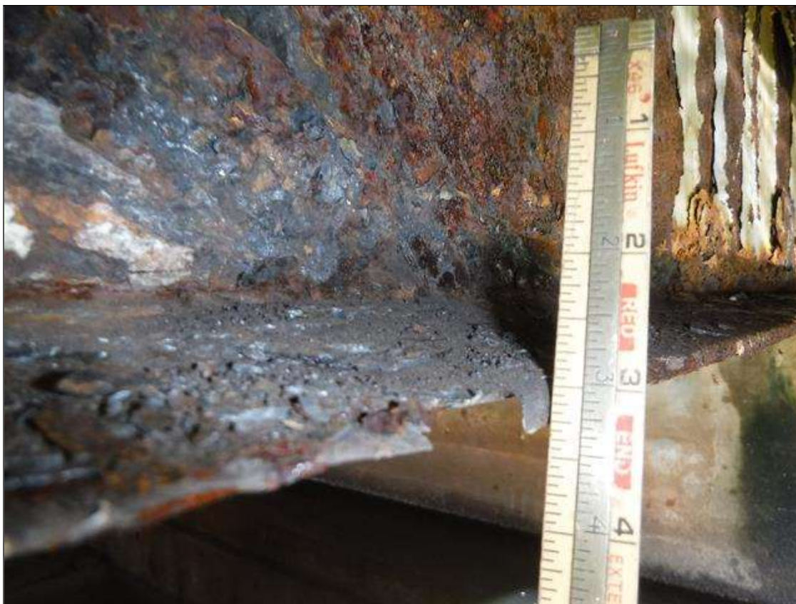
Span 1 Beam 9: SECTION LOSS BOTTOM FLANGE BENT 1 - 100 % 1 IN WIDE X 2 FOOT LONG , 5/16 IN REMAINING WEB SECTION LOSS IN MIDSPAN TO BENT 1 IN BOTTOM FLANGE WITH 1" DIAMETER HOLE IN WEB 6' FROM BENT 1 1/8" PITTING IN WEB FULL HEIGHT. PRIORITY MAINTENANCE ISSUED
