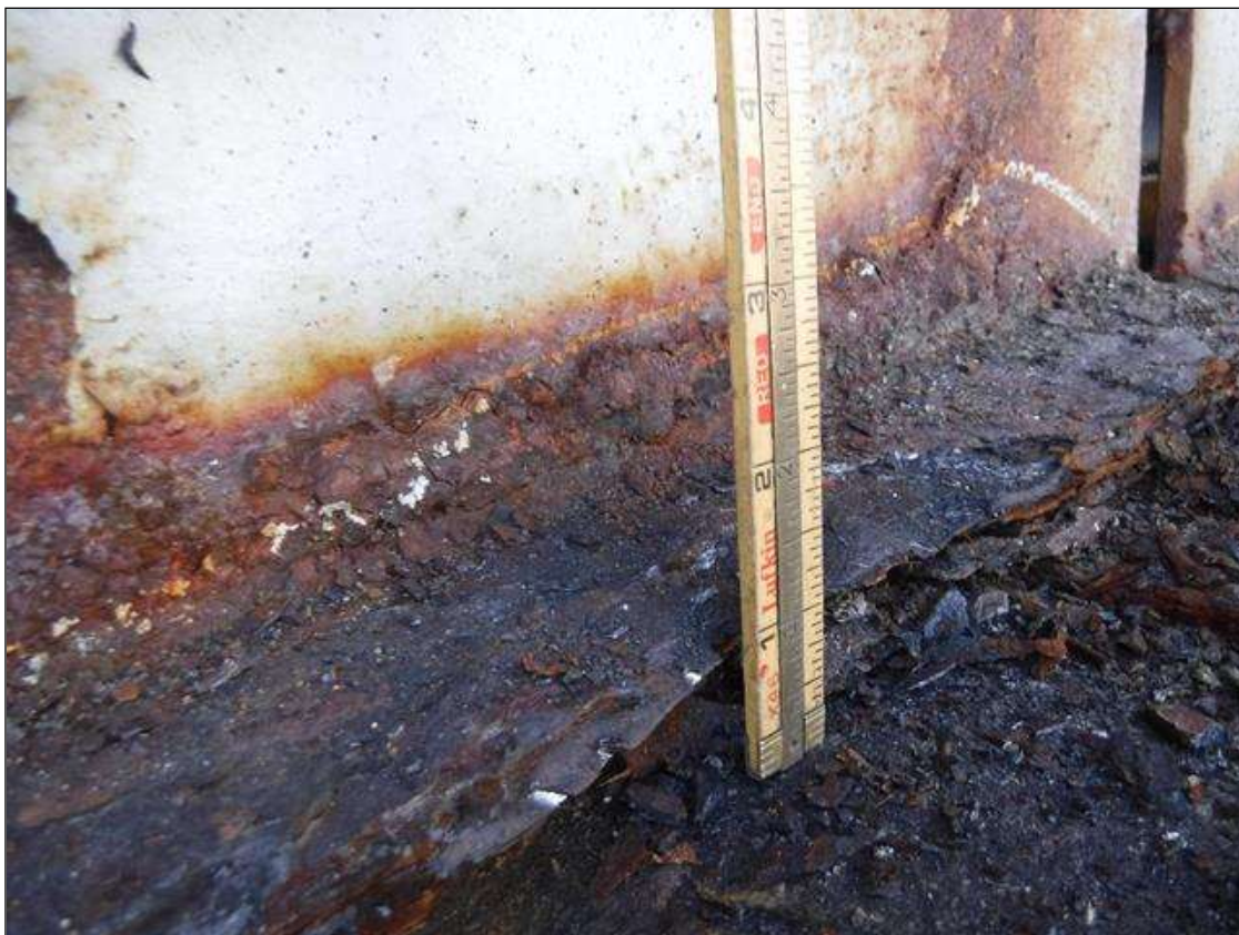
Span 2 Beam 1: SECTION LOSS BOTTOM FLANGE BENT 1 -100 % 1 IN WIDE X 2 FOOT LONG , 1/4 IN REMAINING WEB 4 IN HIGH 2 FOOT LONG PRIORITY MAINTENANCE ISSUED
