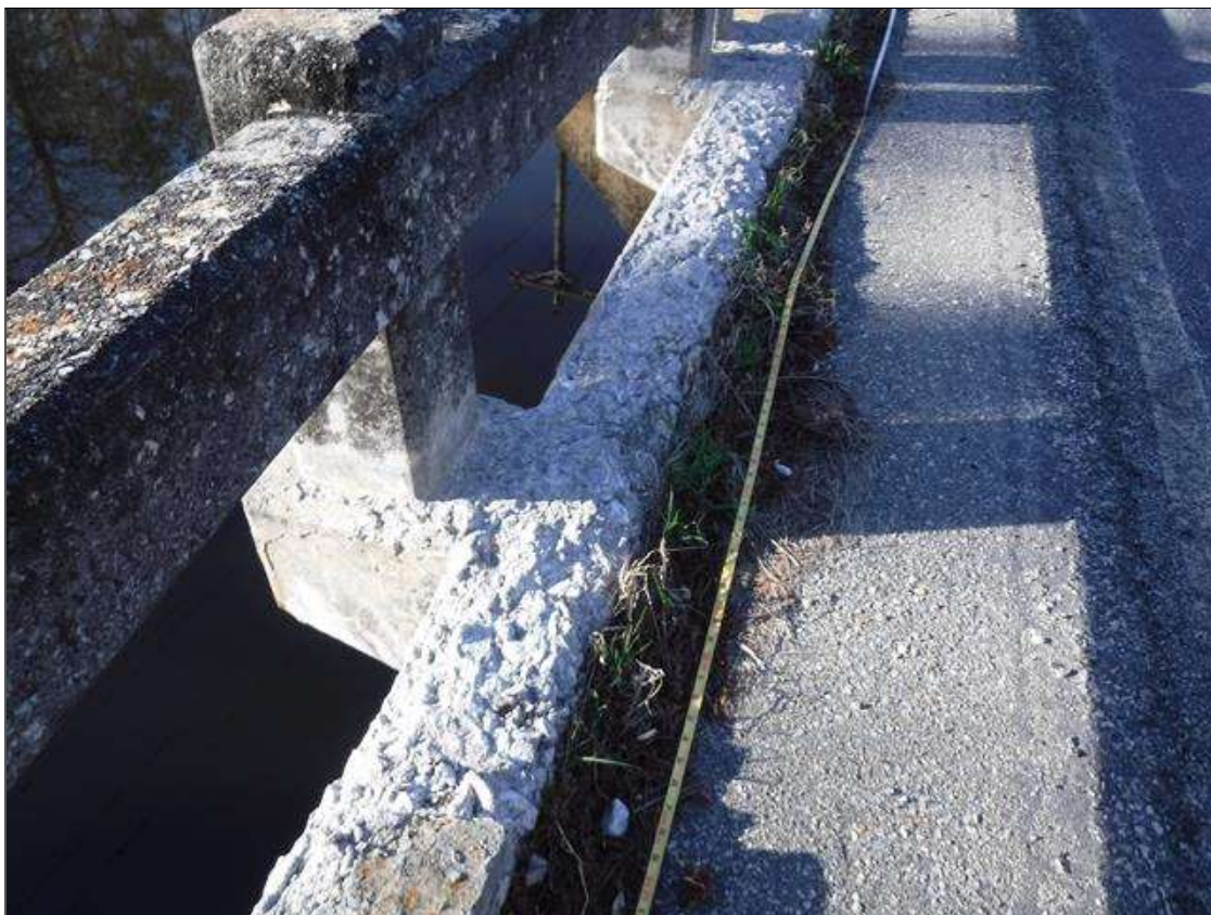
Span 1 Deck: SPALLING IN RIGHT CURB 3 INCH DEEP
