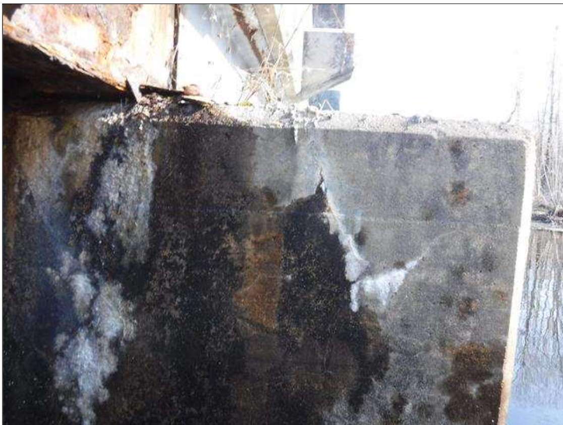
Bent 1 Cap 1: EFFLO IN FACE OF CAP
