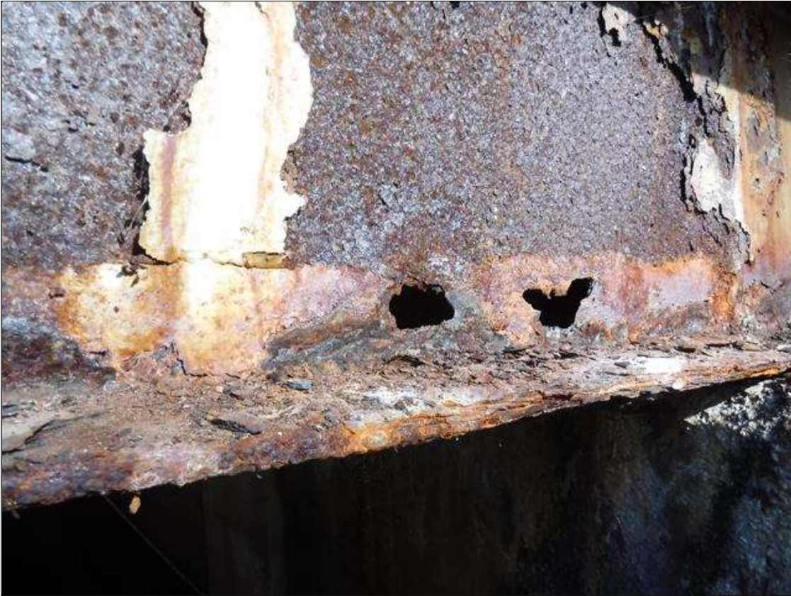
Span 1 Beam 10: SECTION LOSS EDGE BOTTOM FLANGE AT BENT 1 - 100 % 1 IN WIDE X 2 FOOT LONG WITH 3/16 IN REMAINING IN MIDDLE, 5/16 IN REMAINING WEB 4 IN HIGH (2) 2" DIAMETER HOLES IN WEB AREA 2' FROM BENT 1 PRIORITY MAINTENANCE ISSUED
