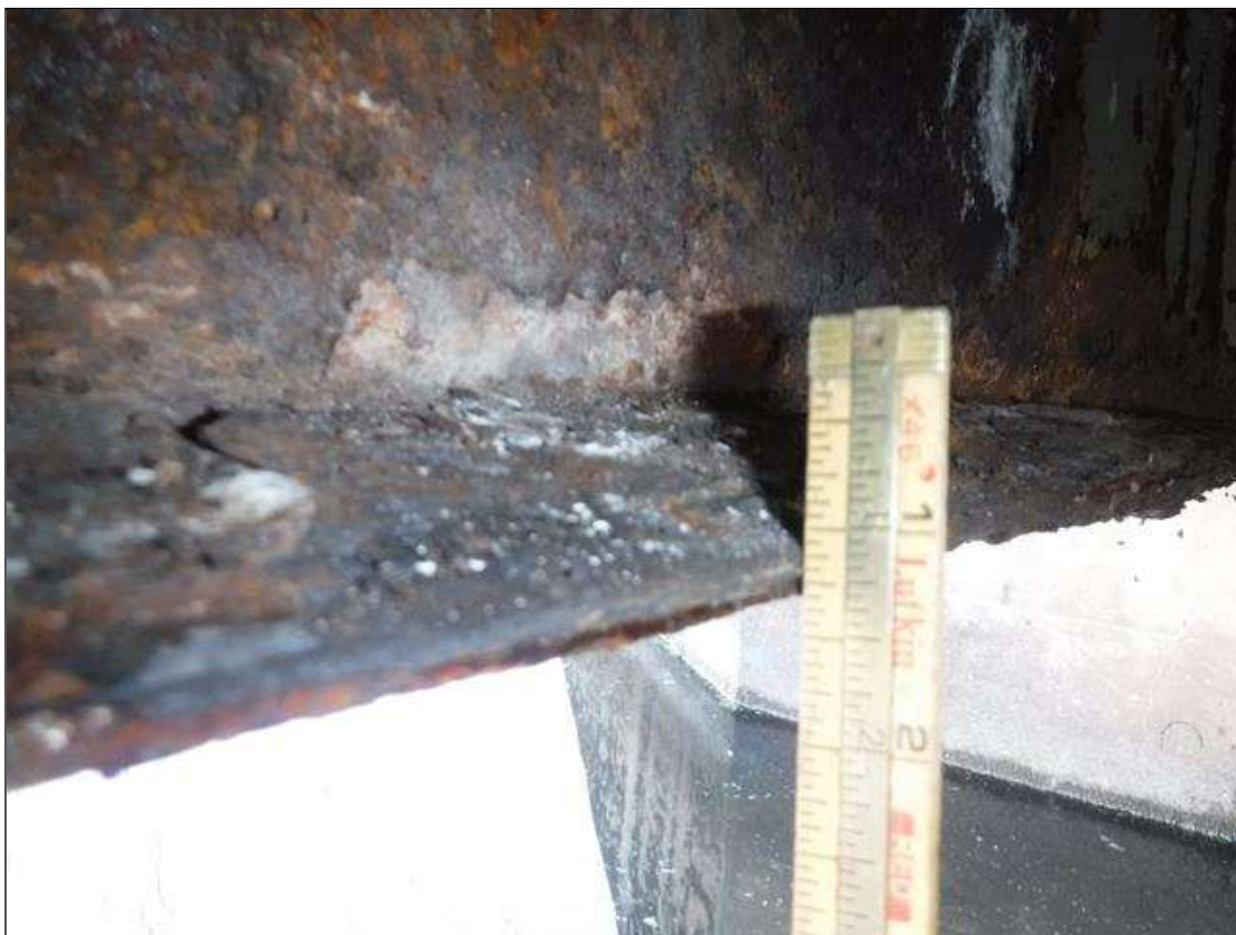
Span 2 Beam 1: SECTION LOSS BOTTOM FLANGE 3/16 IN REMAINING MIDSPAN TO ABUTMENT 2, 5/16 IN REMAINING IN WEB PRIORITY MAINTENANCE ISSUED
