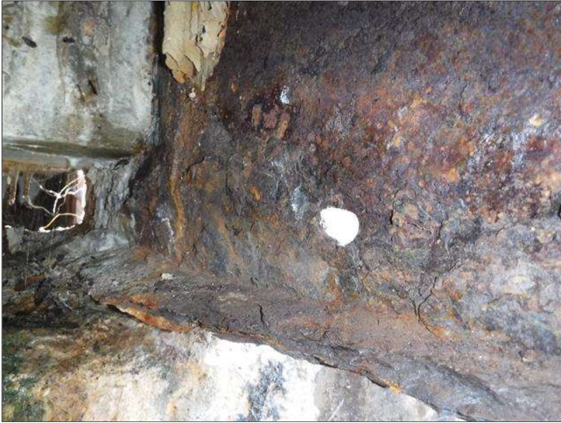
Span 1 Beam 10: SECTION LOSS EDGE BOTTOM FLANGE AT BENT 1 - 100 % 1 IN WIDE X 2 FOOT LONG WITH 3/16 IN REMAINING IN MIDDLE, 5/16 IN REMAINING WEB 4 IN HIGH (2) 2" DIAMETER HOLES IN WEB AREA 2' FROM BENT 1 PRIORITY MAINTENANCE ISSUED
