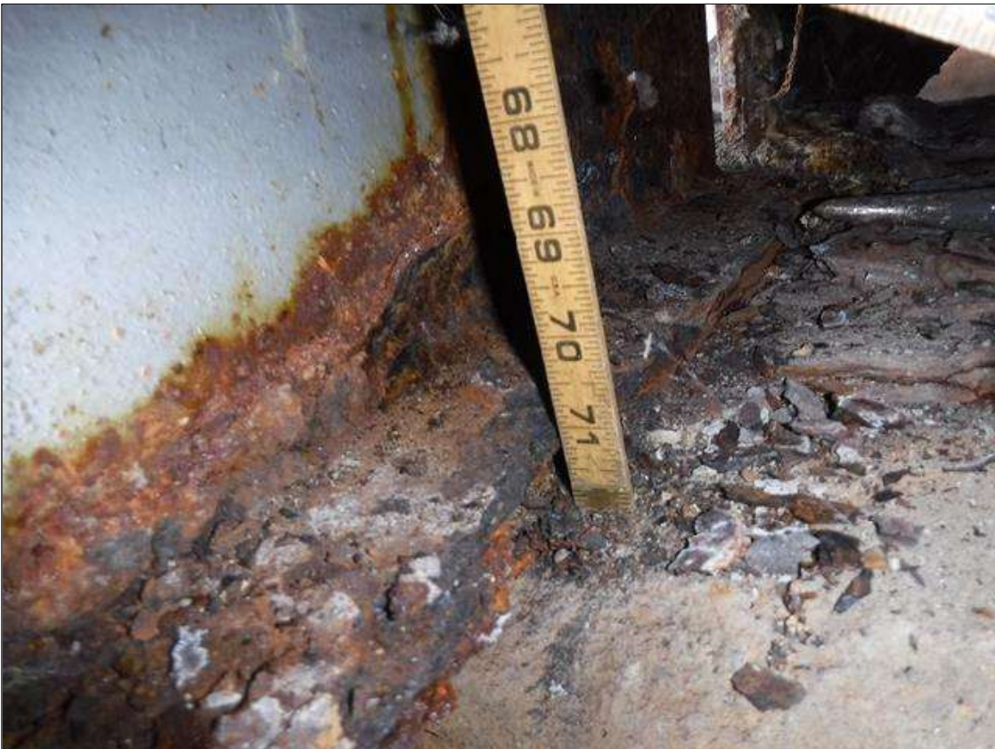
Span 1 Beam 1: SECTION LOSS 100 % 1/2 IN WIDE X 1 FOOT LONG BOTTOM FLANGE BENT 1 REAMINDER DOWN TO KNIFE EDGE, WEB 5/16 IN REMAINING 2 IN HIGH PRIORITY MAINTENANCE ISSUED
