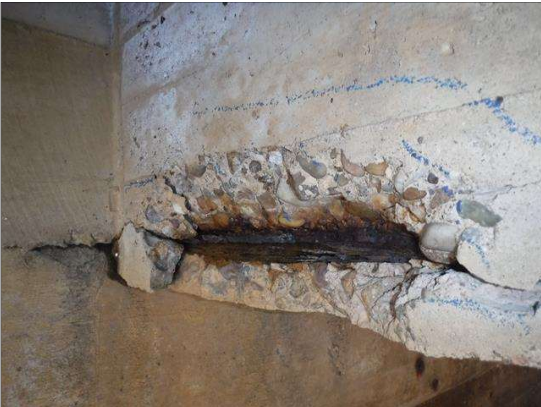
Span 1 Beam 5: SURFACE RUST ON EXPOSED BEAM AT SPALLED COATING
