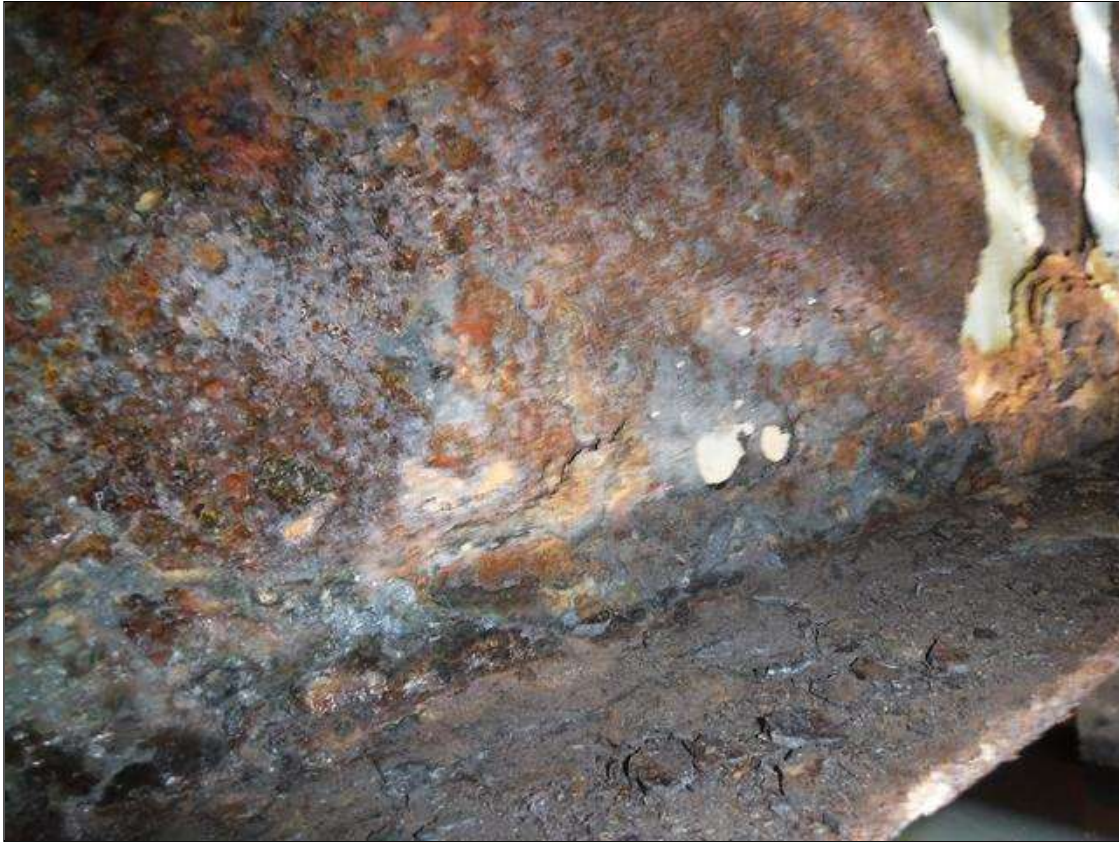
Span 1 Beam 9: SECTION LOSS BOTTOM FLANGE BENT 1 - 100 % 1 IN WIDE X 2 FOOT LONG , 5/16 IN REMAINING WEB SECTION LOSS IN MIDSPAN TO BENT 1 IN BOTTOM FLANGE WITH 1" DIAMETER HOLE IN WEB 6' FROM BENT 1 1/8" PITTING IN WEB FULL HEIGHT. PRIORITY MAINTENANCE ISSUED
