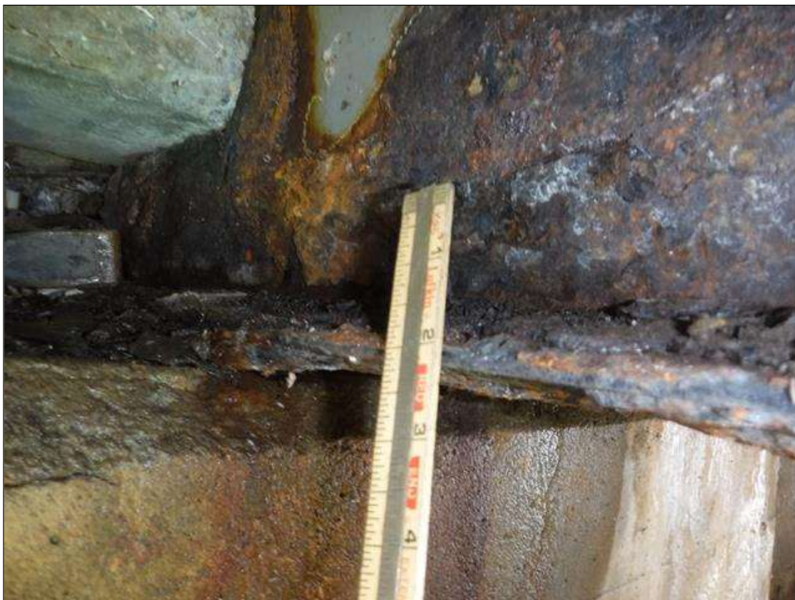
Span 2 Beam 9: SECTION LOSS 1/4 IN REMAINING BOTTOM FLANGE 4 FOOT LONG AT BENT 1, 5/16 IN REMAINING WEB 8 IN HIGH X 3 FOOT PRIORITY MAINTENANCE ISSUED
