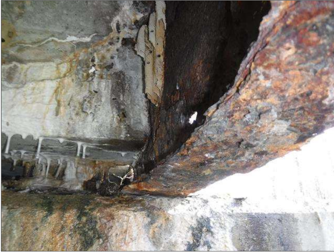
Span 1 Beam 10: SECTION LOSS EDGE BOTTOM FLANGE AT BENT 1 - 100 % 1 IN WIDE X 2 FOOT LONG WITH 3/16 IN REMAINING IN MIDDLE, 5/16 IN REMAINING WEB 4 IN HIGH (2) 2" DIAMETER HOLES IN WEB AREA 2' FROM BENT 1 PRIORITY MAINTENANCE ISSUED
