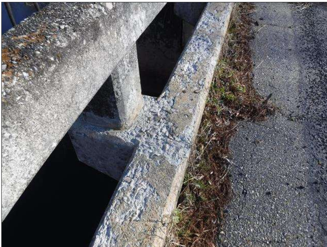
Span 2 Deck: SPALLING 1/2 IN DEEP TOP LEFT CURB
