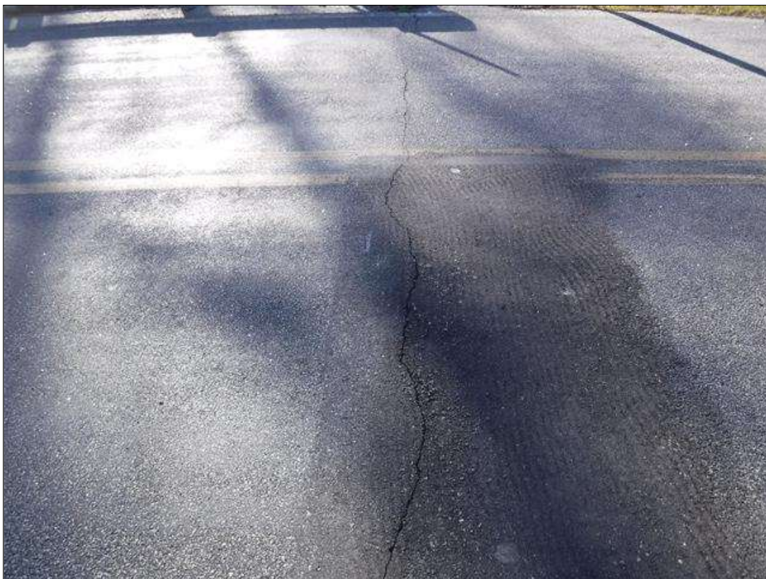
Span 1 Wearing Surface: TRANSVERSE CRACKING END BENT 1
