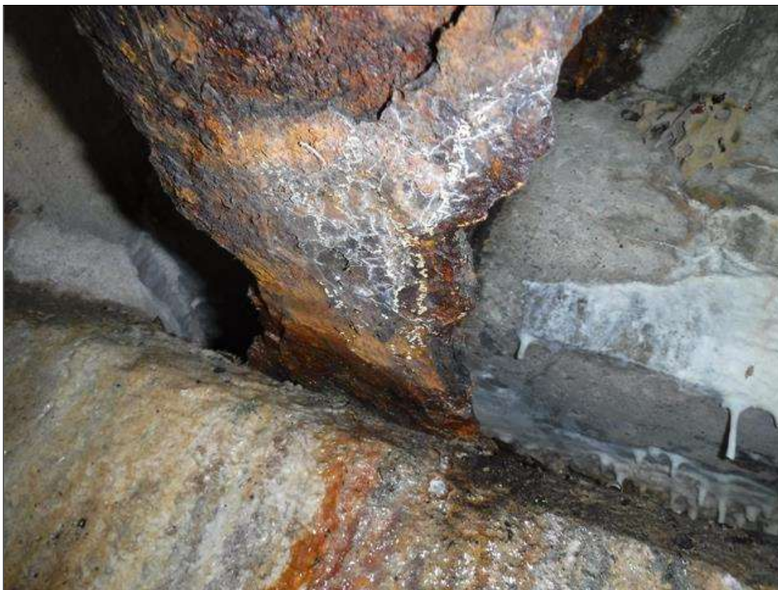
Span 1 Beam 9: SECTION LOSS BOTTOM FLANGE BENT 1 - 100 % 1 IN WIDE X 2 FOOT LONG , 5/16 IN REMAINING WEB SECTION LOSS IN MIDSPAN TO BENT 1 IN BOTTOM FLANGE WITH 1" DIAMETER HOLE IN WEB 6' FROM BENT 1 1/8" PITTING IN WEB FULL HEIGHT. PRIORITY MAINTENANCE ISSUED
