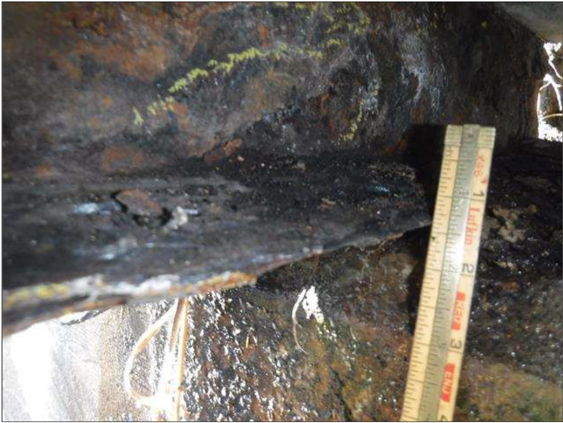
Span 2 Beam 10: SECTION LOSS BOTTOM FLANGE BENT 1 DOWN TO KNIFE EDGE , WEB 5/16 IN REMAINING 4 IN HIGH X 3 FOOT PRIORITY MAINTENANCE ISSUED
