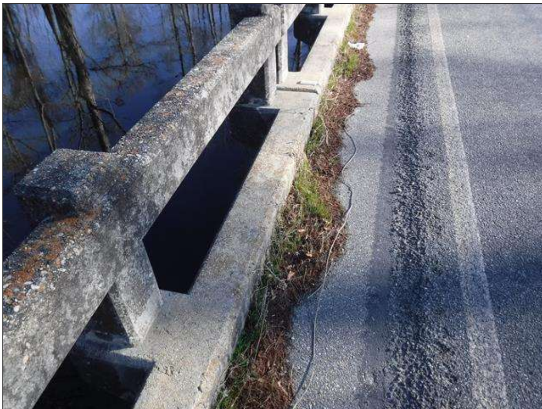
DEBRIS VEGETATION ALONG CURBS
