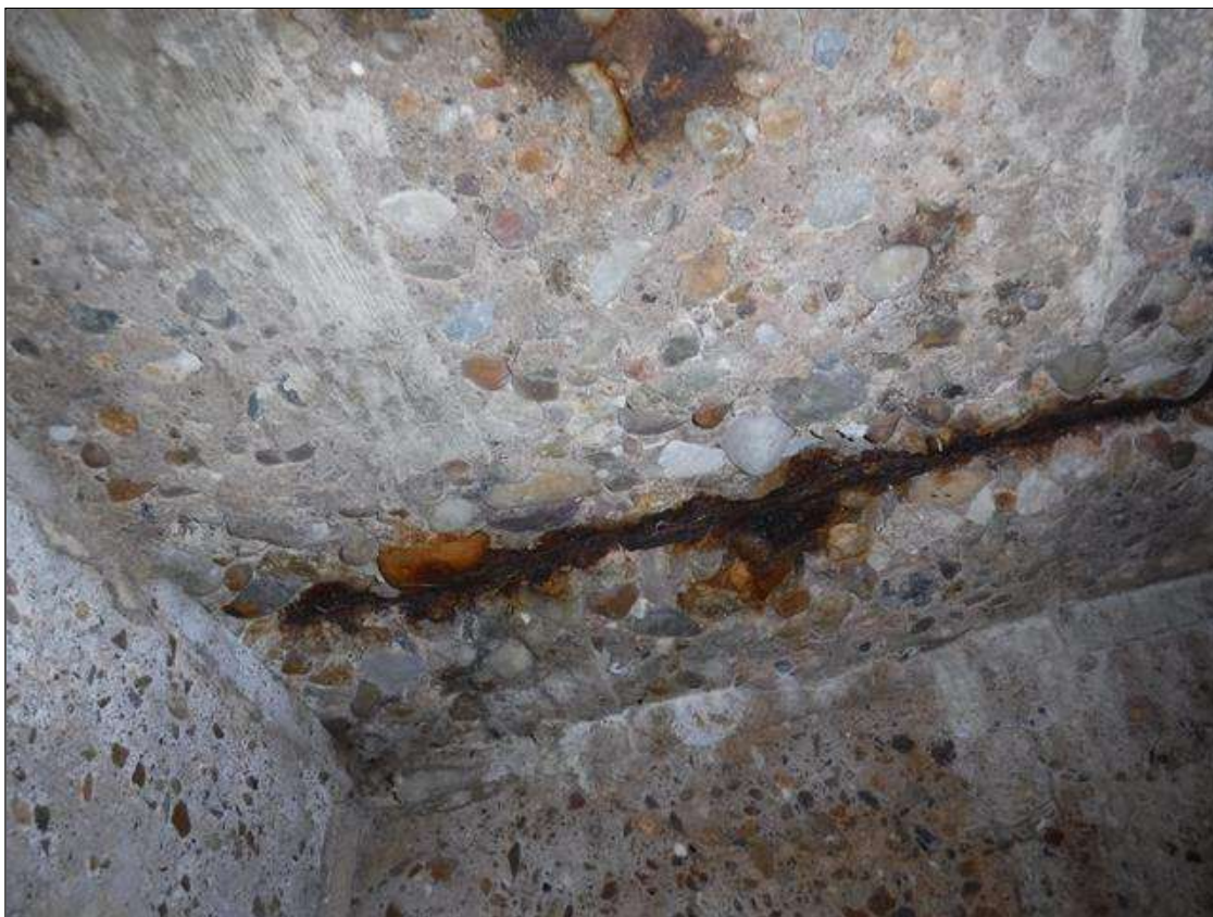
Span 2 Deck: SPALL IN BOTTOM OF DECK UNDER BAY 3 WITH EXPOSED STEEL
