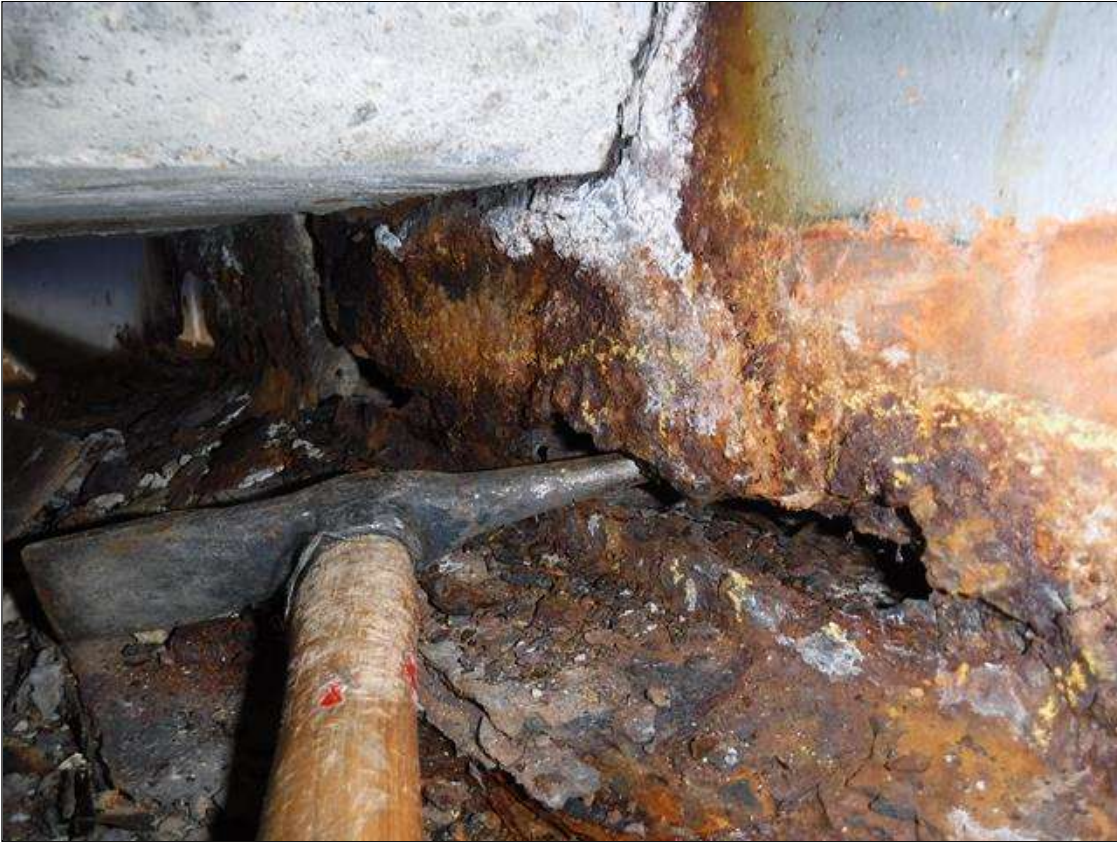
Span 1 Beam 2: SECTION LOSS WEB BENT 1 HOLE 1 IN HIGH X 10 IN LONG , SECTION LOSS 100 % EDGE BOTTOM FLANGE 2 IN WIDE X 2 FOOT LONG PRIORITY MAINTENANCE ISSUED
