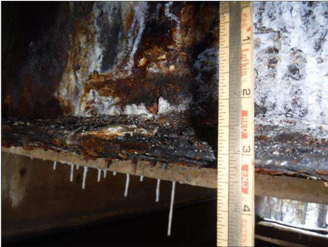
Span 2 Beam 2: 3/16" REMAINING SECTION LOSS BOTTOM FLANGE ABUTMENT 2 - 1/4 IN REMAINING WEB 3/4 IN REMAINING FULL HEIGHT 8 FOOT LONG PRIORITY MAINTENANCE ISSUED
