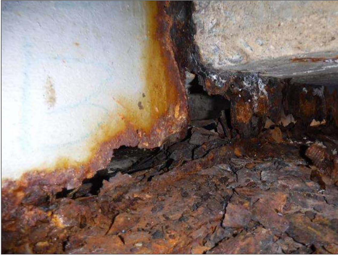
Span 2 Beam 2: HOLE IN WEB AT BENT 1 - 3 IN HIGH X 14 IN LONG REMAINDER 1/8 IN REMAINING 1 FOOT LONG, BOTTOM FLANGE 100 % SECTION LOSS 3/4 IN WIDE X 2 FOOT LONG , DOWN TO KNIFE EDGE 1/6 IN REMAINING AT EDGE 4 FOOT LONG PRIORITY MAINTENANCE ISSUED
