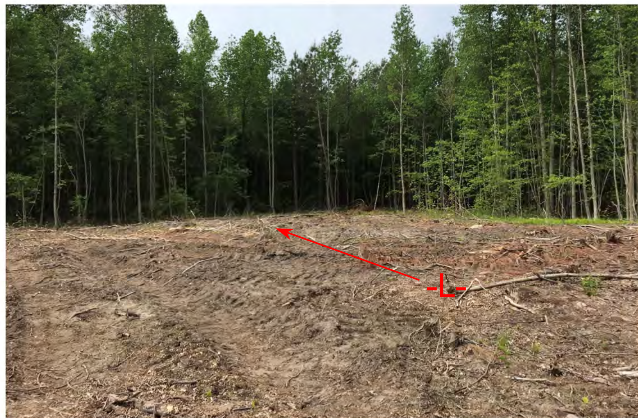
NORTH APPROACH TO END BENT 1, ALONG -L- ALIGNMENT NORTH OF CSX RR, LOOKING SOUTHWEST
