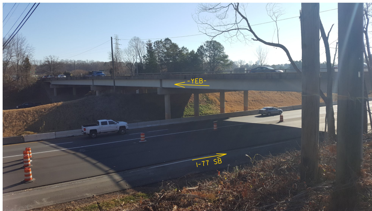
Photo No. 2: View at existing Bent 1 looking east (upstation) on -YEB- (SR 2136)
