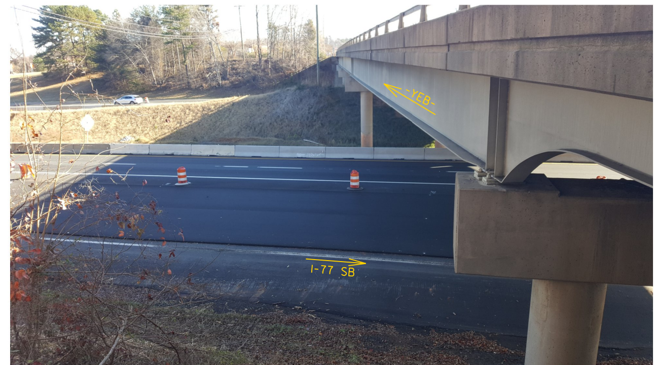
Photo No. 3: View at End Bent 1 looking east (upstation) on -YEB- (SR 2136)
